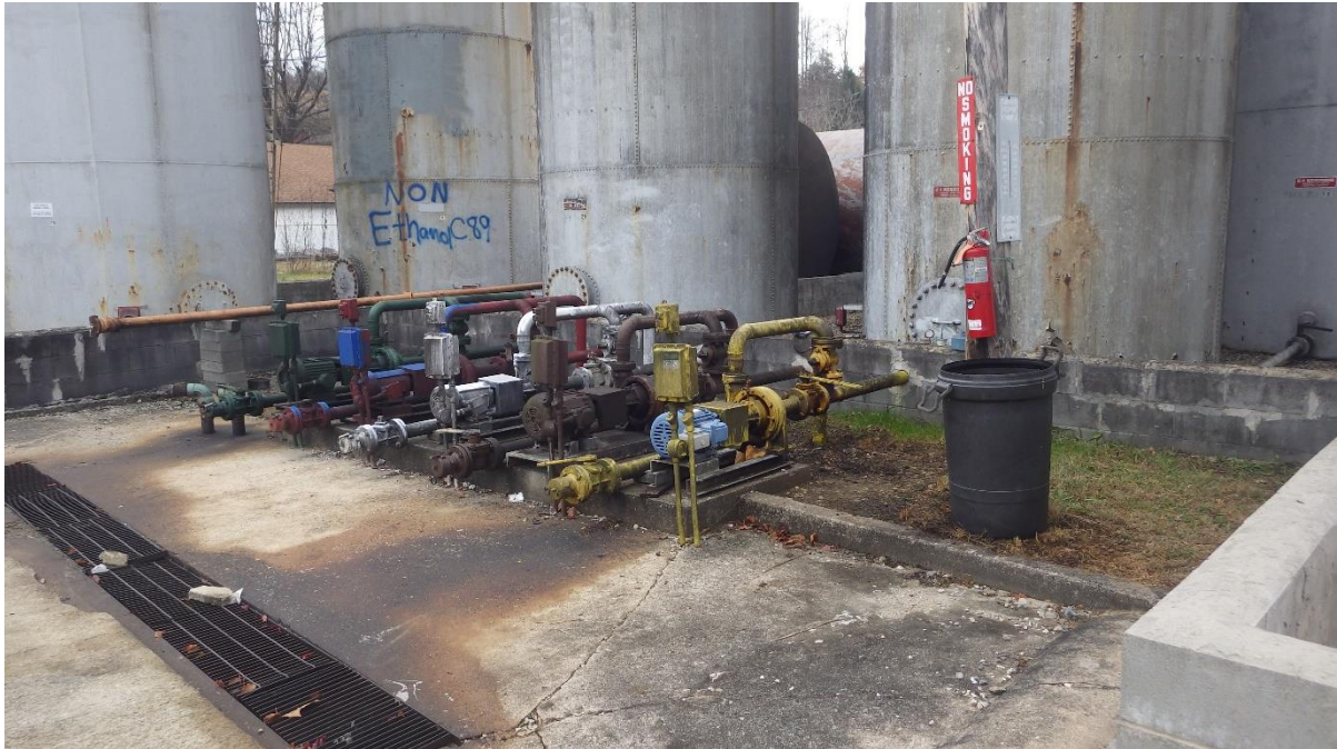
ASTs refill area with release catch basin.
