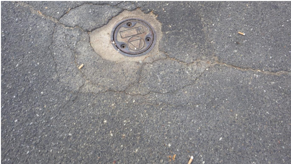
Monitoring well (not secured)
