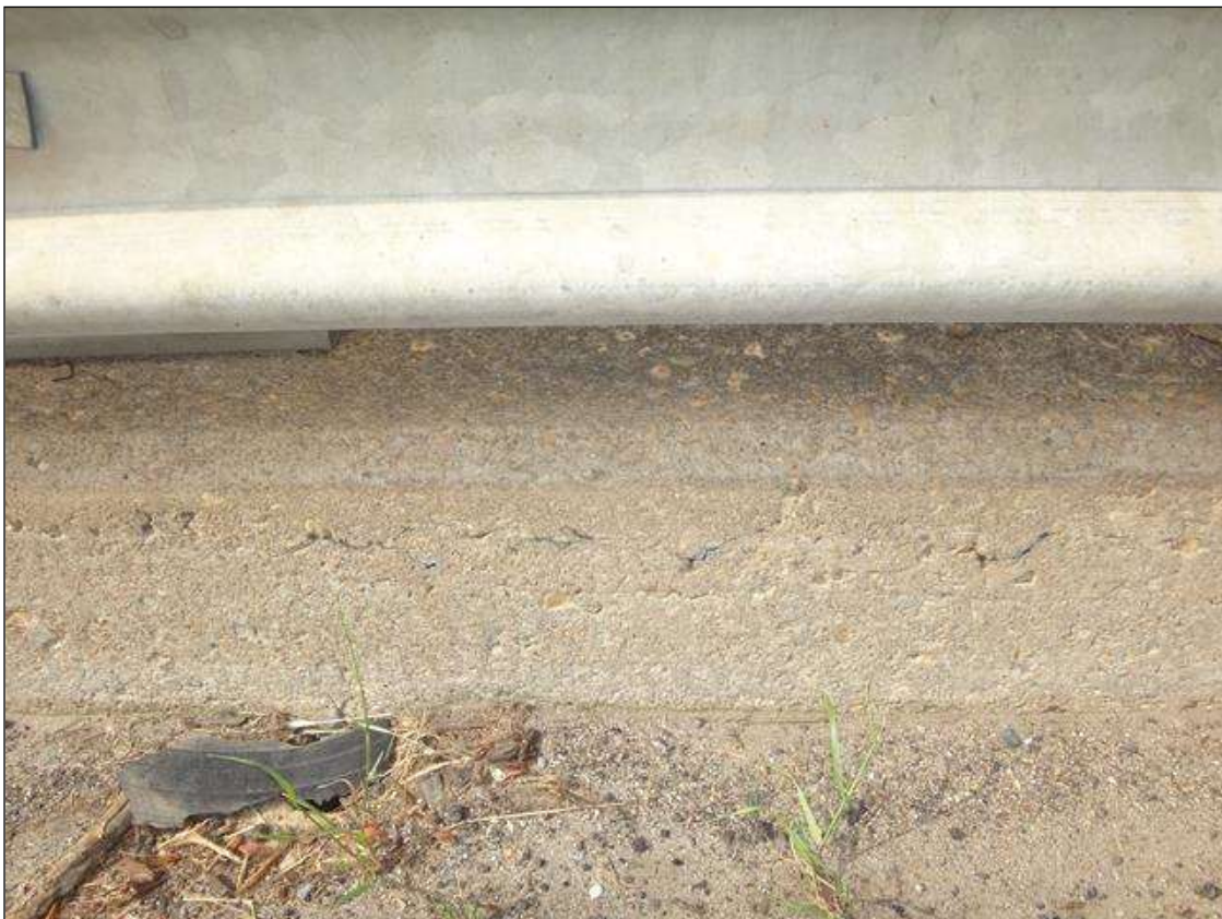
SPAN 5 SOUTH RAIL PARAPET, HORIZONTAL CRACK (3FT X 1/16IN)
