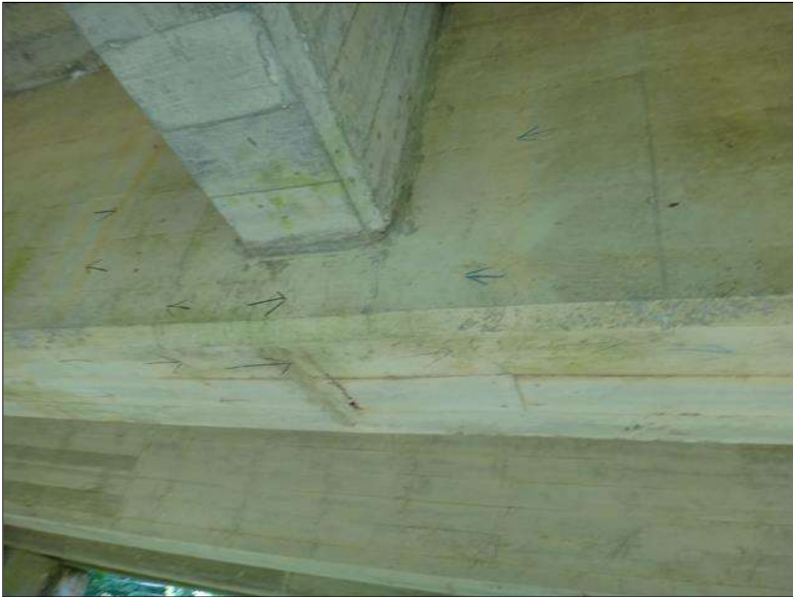
SPAN 2 BEAM 2 AT MIDSPAN, MULTIPLE TRANSVERSE CRACKS (FULL WIDTH X HAIRLINE) EXTEND UP BOTH SIDES WITH ADJACENT MAP CRACKING
