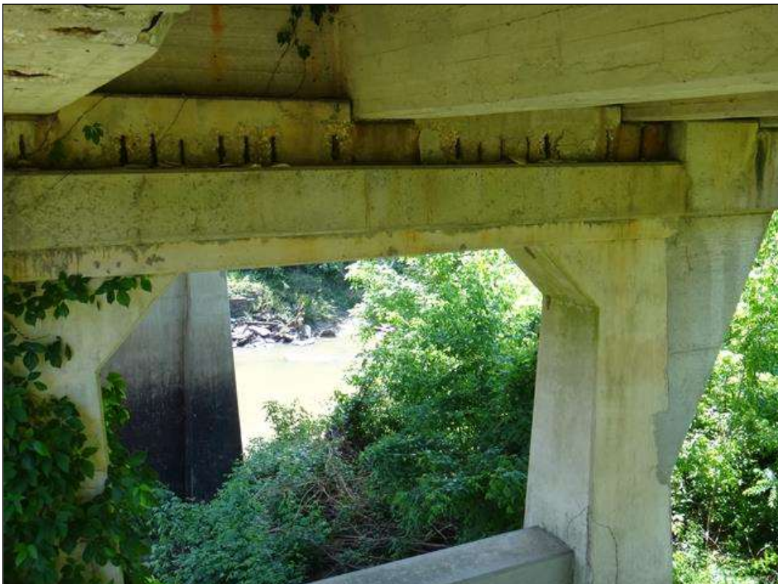
(PM) BENT 6 CAP WEST FACE, MULTIPLE SPALLS (UP TO 20IN X 12IN)
