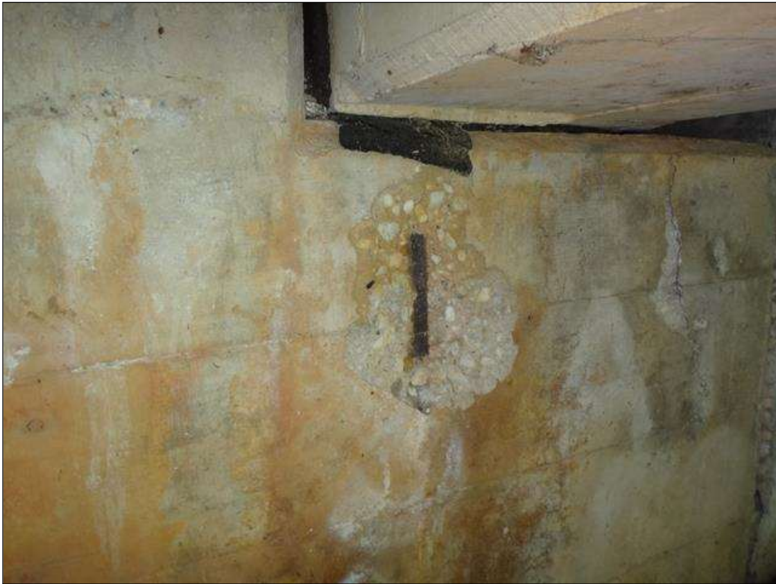
(PM) END BENT 2 CAP WEST FACE BELOW BEAM 4, SPALL (8IN X 6IN X 1IN DEEP) WITH EXPOSED RUSTED REBAR
