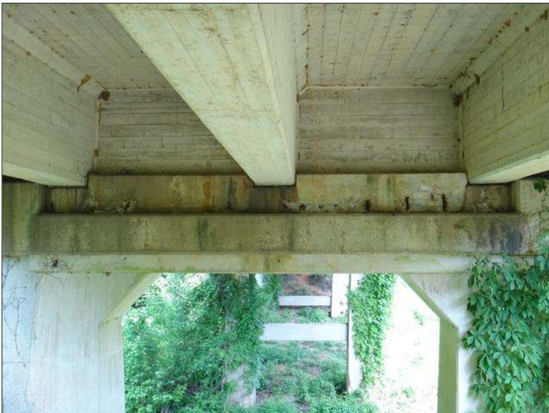
(PM) BENT 3 CAP EAST FACE, MULTIPLES SPALLS (UP TO 3FT X 10IN X 2IN DEEP) WITH EXPOSED RUSTED REBAR, SECTION LOSS (NO MEASURABLE LOSS)
