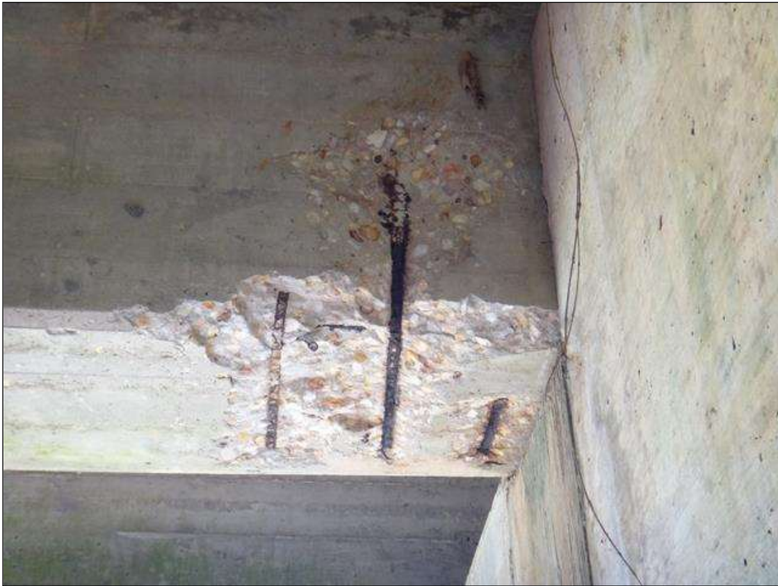
(PM) SPAN 1 BEAM 2 AT BENT 1, SPALL (24IN X 20IN X 2IN DEEP) WITH EXPOSED RUSTED REBAR, SECTION LOSS ON SECONDARY (UP TO 50%)
