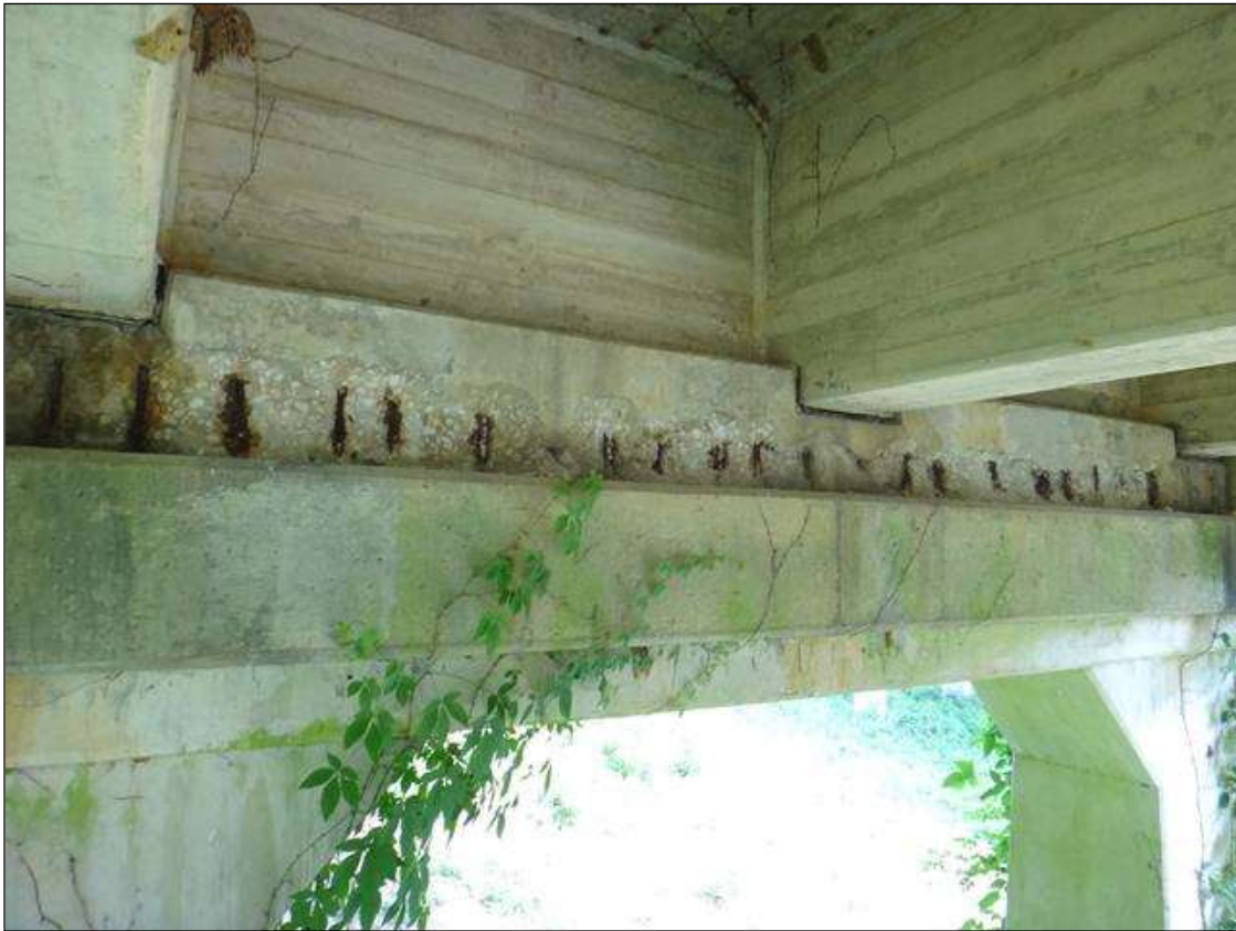
(PM) BENT 2 CAP EAST FACE, SPALL (17FT X 12IN X 2IN) WITH EXPOSED RUSTED REBAR, SECTION LOSS (NO MEASURABLE LOSS), DELAMINATION (FULL WIDTH X 15IN)
