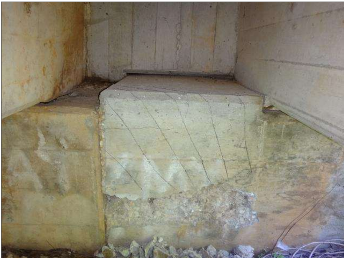
END BENT 2 BAY 4 CAP WEST AND TOP FACE, SPALL (3FT X 1FT X 3IN DEEP), DELAMINATION (3FT X 2FT)
