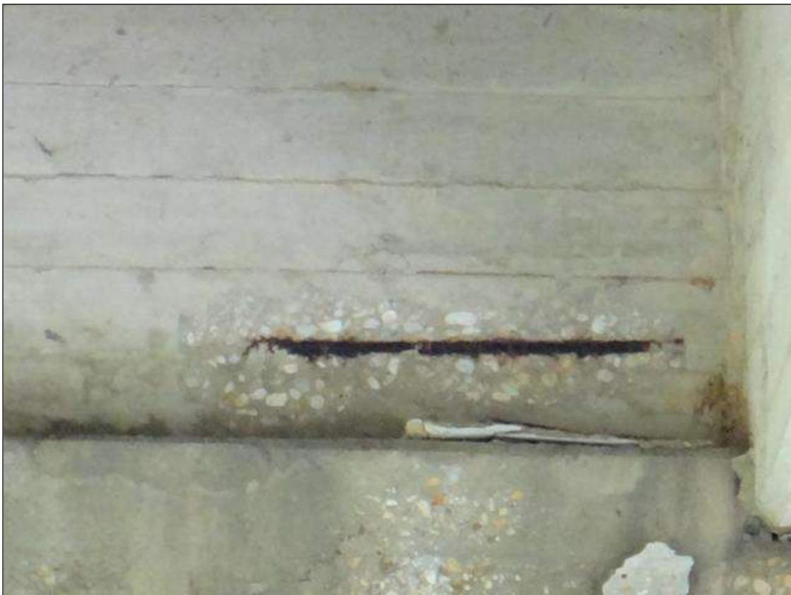
SPAN 6 BENT 5 END DIAPHRAGM AT BAY 4, SPALL (20IN X 5IN X 1IN DEEP) WITH EXPOSED RUSTED REBAR
