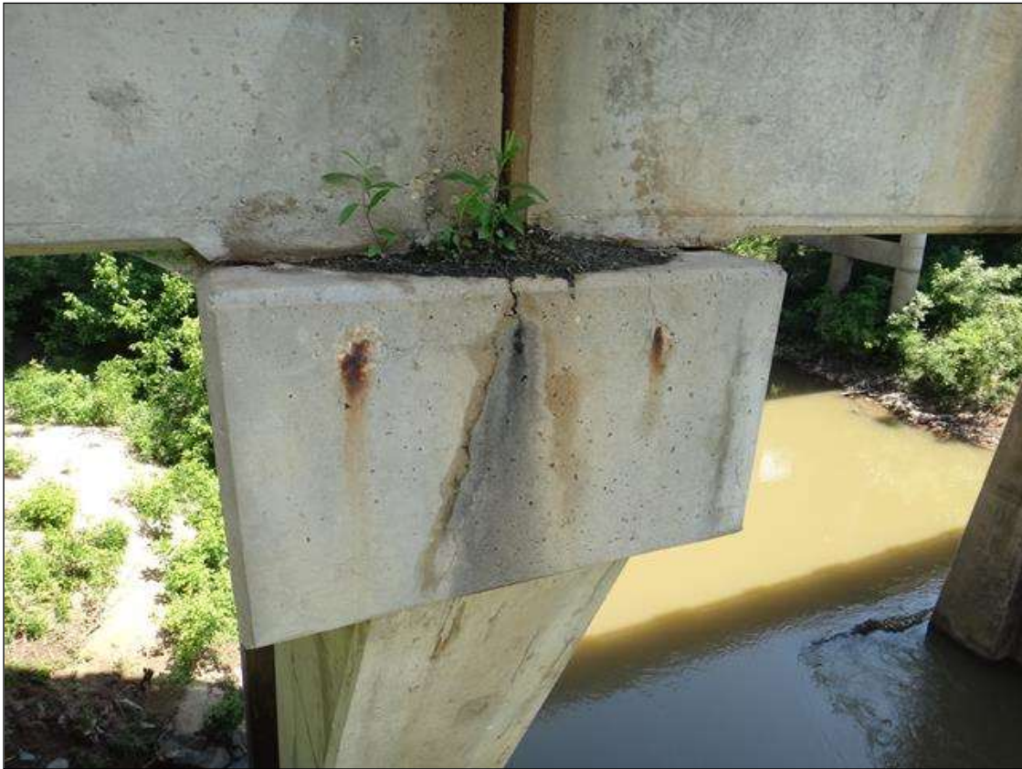
(PM) BENT 7 CAP AT SOUTH END, TWO (2) POPOUTS (3IN X 1/2IN) WITH EXPOSED RUSTED REBAR, THREE (3) VERTICAL CRACKS (FULL HEIGHT X HAIRLINE), AND DEBRIS
