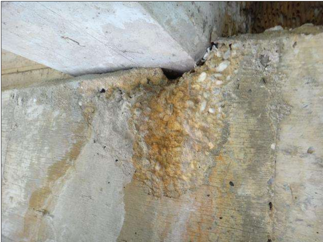
BENT 7 CAP EAST FACE BELOW BEAM 2, SPALL (16IN X 11IN X 2IN DEEP)
