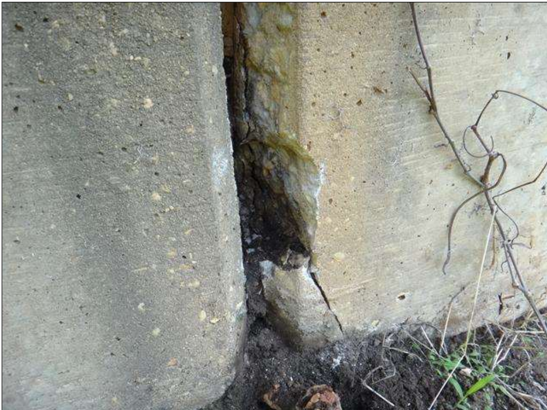
SPAN 5 BEAM 5 SOUTH FACE AT BENT 5, SPALL (12IN X 4IN X 2IN DEEP) WITH ADJACENT DELAMINATION
