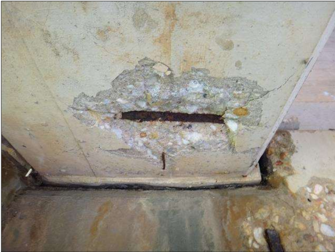
(PM) SPAN 7 BEAM 4 AT BENT 6, SPALL ON BOTTOM FACE (8IN X 6IN X 2IN DEEP) WITH EXPOSED RUSTED REBAR
