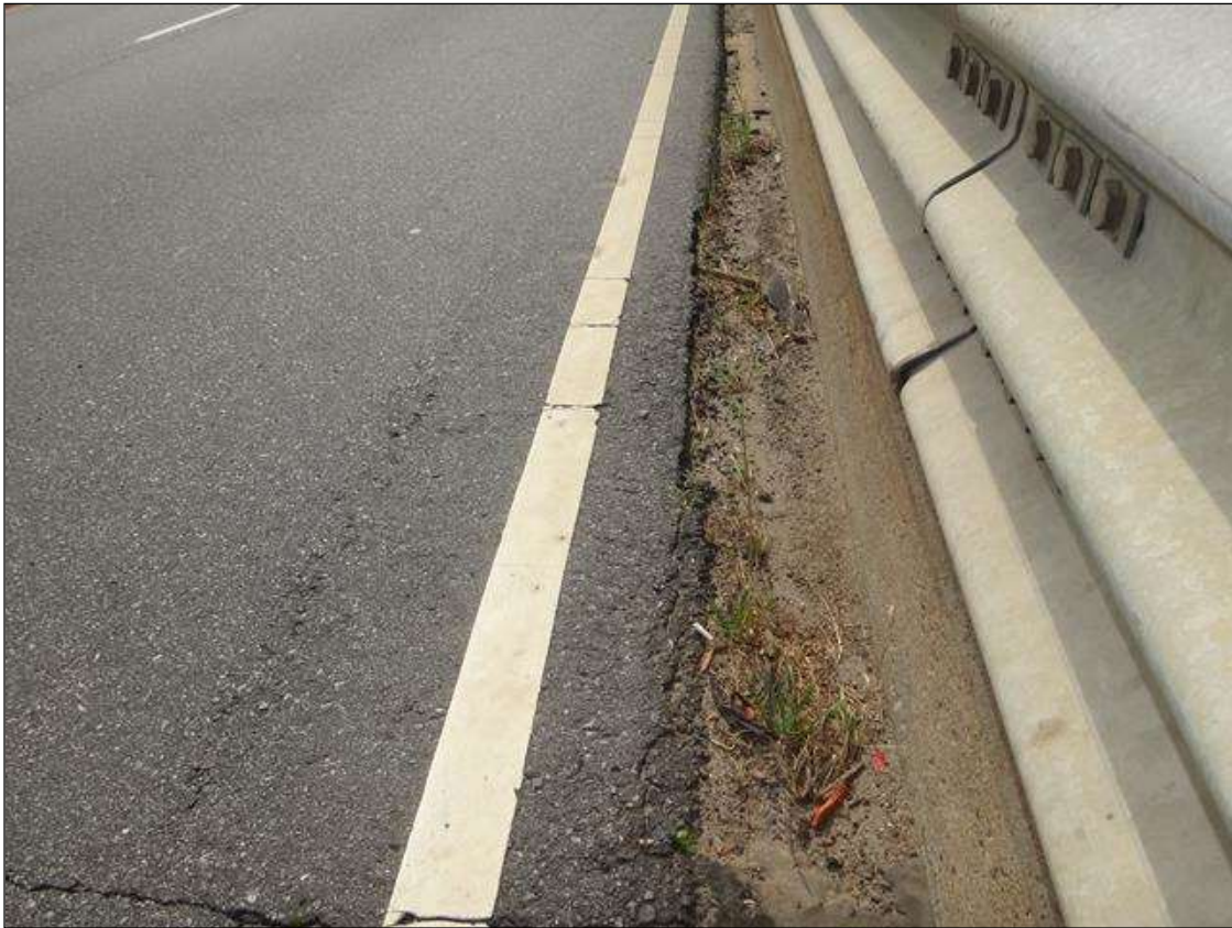
SPAN 4 SOUTH CURB, DEBRIS ACCUMULATION WITH VEGETATION GROWTH (FULL LENGTH X 1FT)
