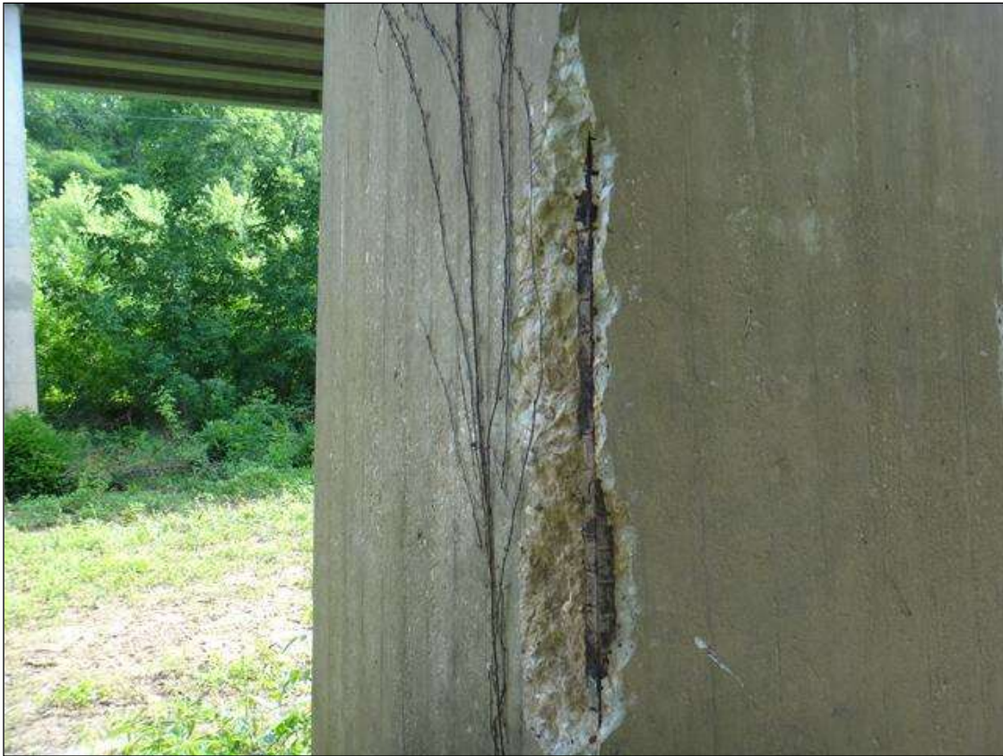
(PM) BENT 4 COLUMN 1 SOUTHWEST CORNER, SPALL (4FT X 8IN X 3IN DEEP) WITH EXPOSED RUSTED REBAR, SECTION LOSS (NO MEASURABLE LOSS)
