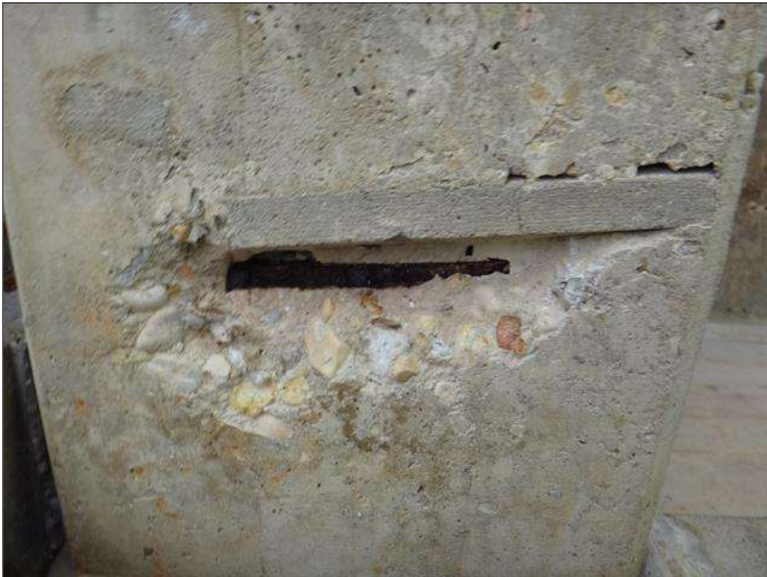
(PM) SPAN 2 BEAM 2 AT BENT 2, SPALL (14IN X 6IN X 2IN DEEP) WITH EXPOSED RUSTED REBAR
