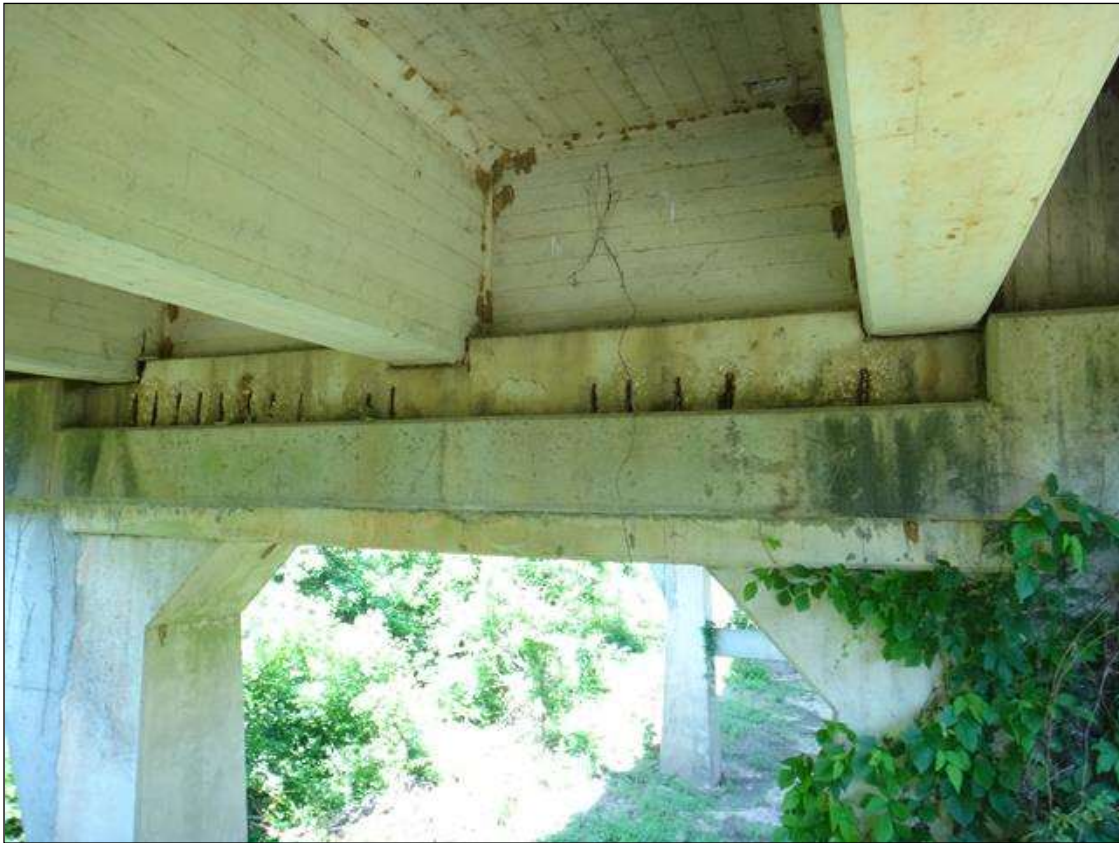
(PM) BENT 6 CAP EAST FACE, MULTIPLE SPALLS/DELAMINATIONS (UP TO 5-1/2FT X 16IN X 2IN) WITH EXPOSED RUSTED REBAR, SECTION LOSS (NO MEASURABLE LOSS)
