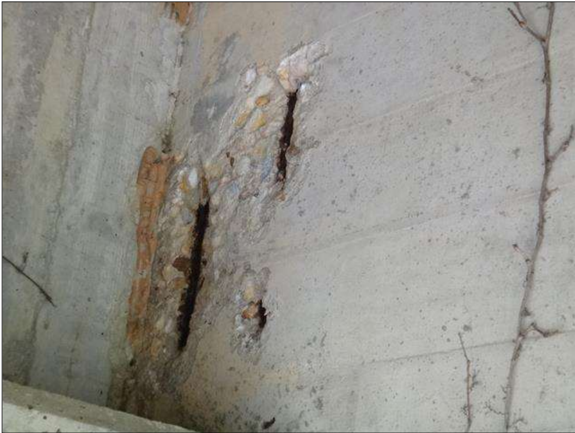
(PM) SPAN 3 BEAM 2 AT BENT 3, THREE (3) SPALLS (UP TO 18IN X 6IN X 1IN DEEP) WITH EXPOSED RUSTED REBAR
