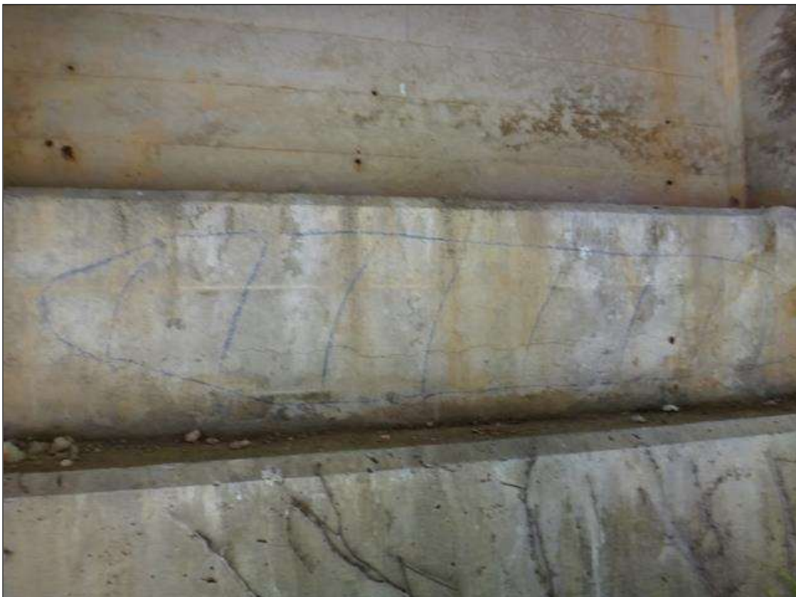
BENT 2 CAP WEST FACE AT BAY 3, DELAMINATION (6FT X 18IN)
