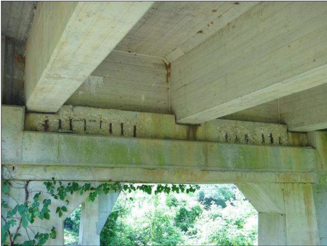
(PM) BENT 5 CAP WEST FACE, TWO (2) SPALLS (6FT X UP TO 20IN X 3IN DEEP) WITH EXPOSED RUSTED REBAR, SECTION LOSS (NO MEASURABLE LOSS)
