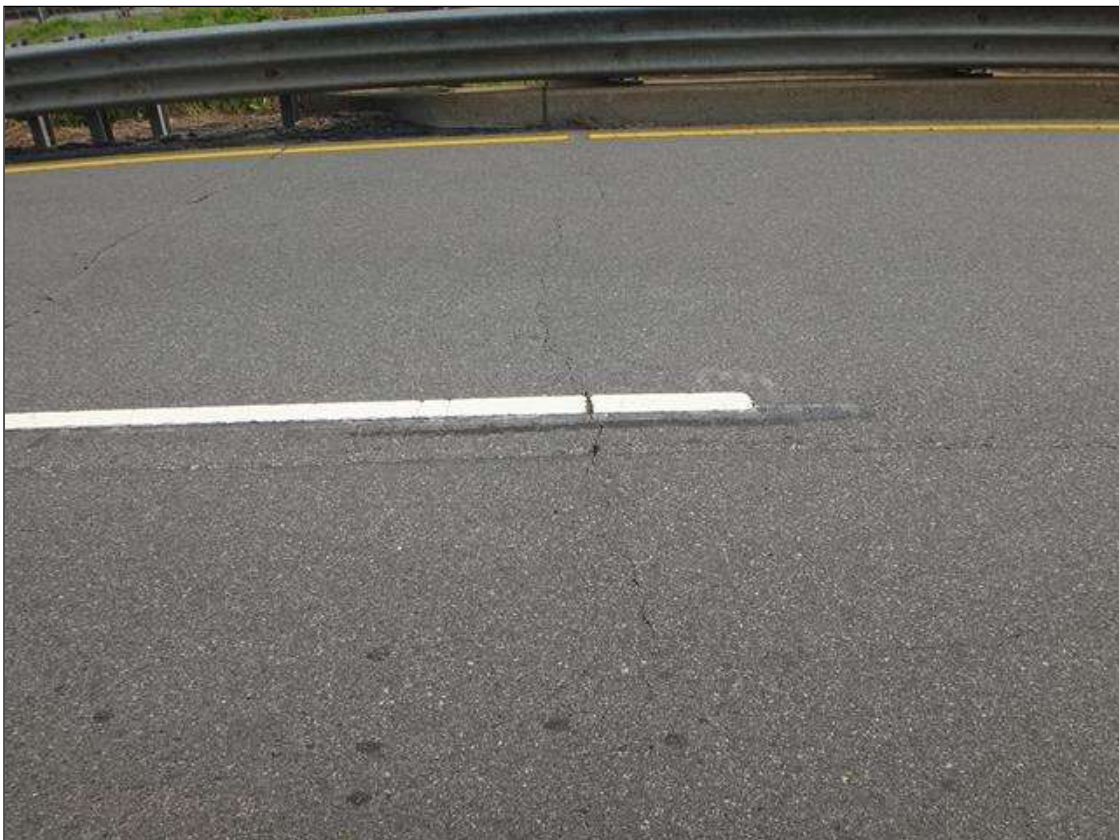
ASPHALT WEARING SURFACE OVER END BENT 1, TRANSVERSE CRACK (FULL WIDTH X UP TO 1/4IN)
