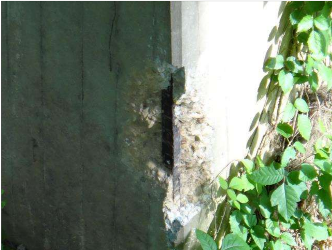
(PM) BENT 2 COLUMN 1 SOUTHEAST CORNER, SPALL (30IN X 12IN X 2IN DEEP) WITH EXPOSED RUSTED REBAR
