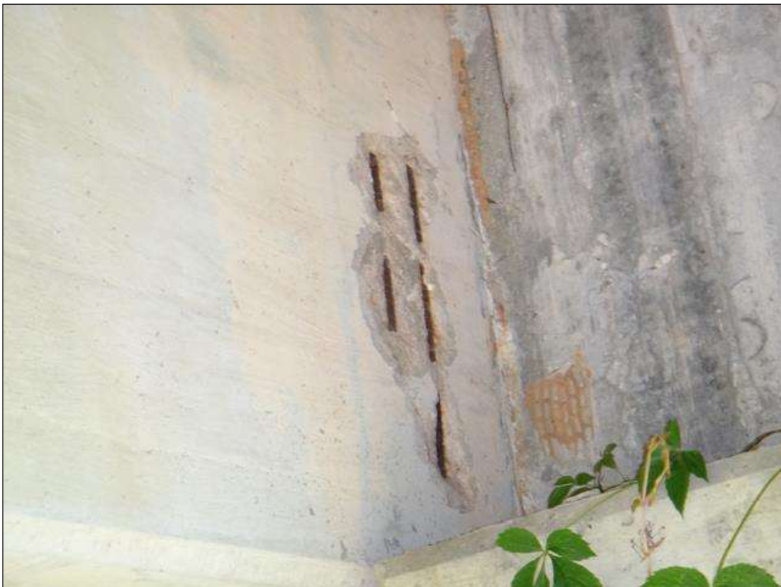
(PM) SPAN 4 BEAM 2 AT BENT 3, SPALL (18IN X 8IN X 1IN DEEP) WITH EXPOSED RUSTED REBAR
