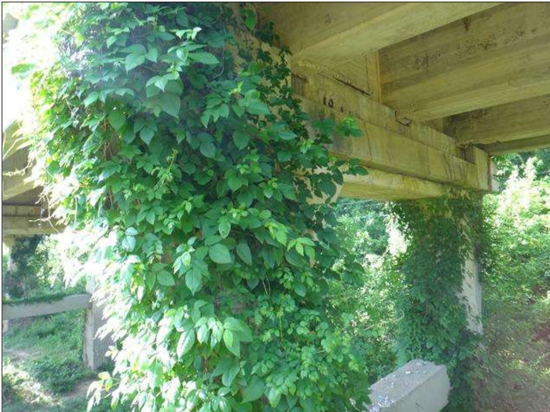
BENT 2 CAP AND COLUMN, VEGETATION GROWTH
