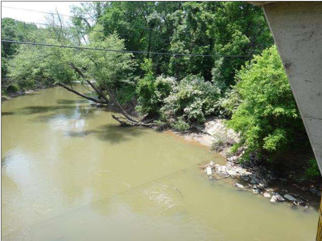
SOUTHWEST STREAMBANK, EROSION WITH DISPLACED SLOPE PROTECTION AND EXPOSED TREE ROOTS
