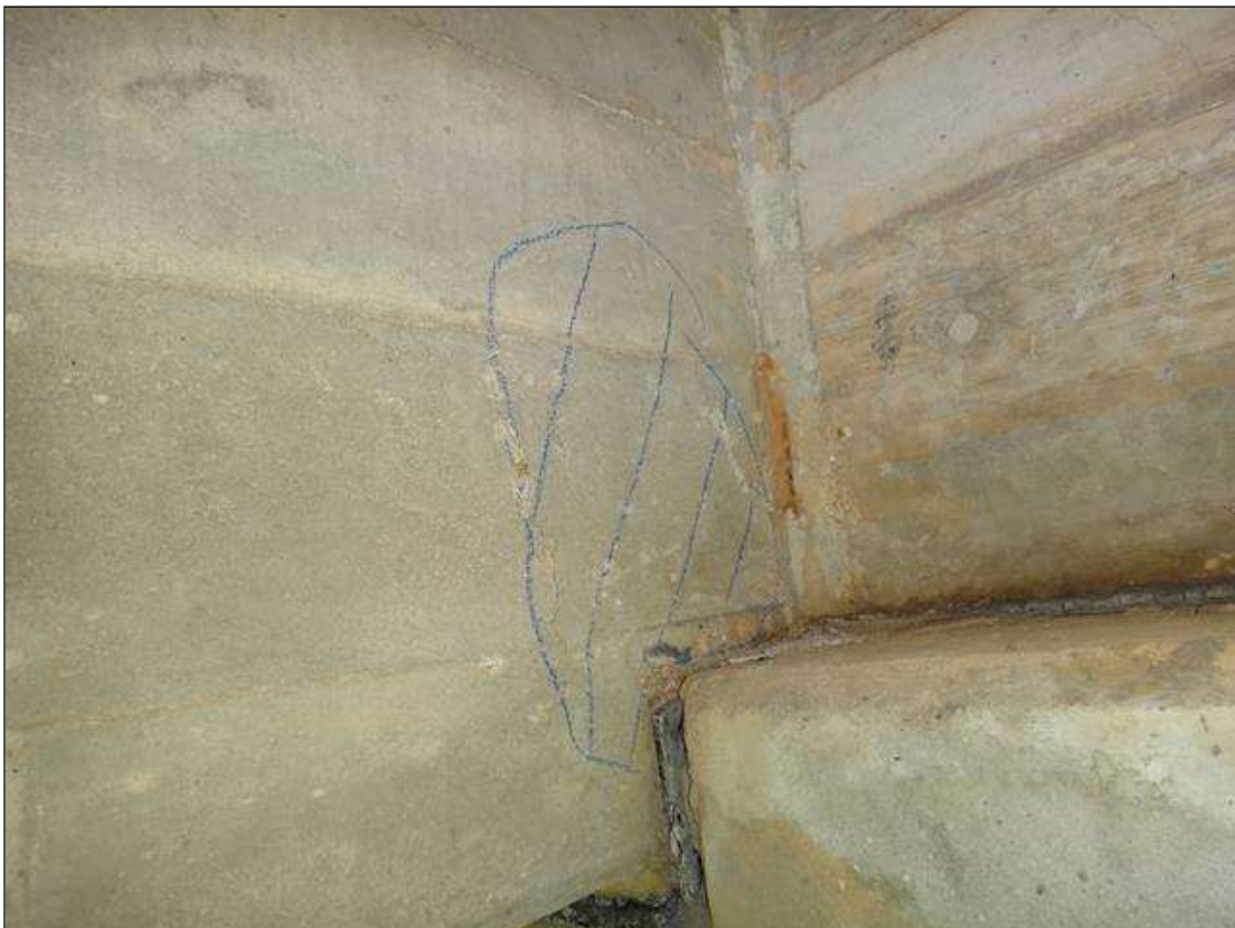
SPAN 3 BEAM 3 NORTH FACE AT BENT 2, DELAMINATION (14IN X 10IN)
