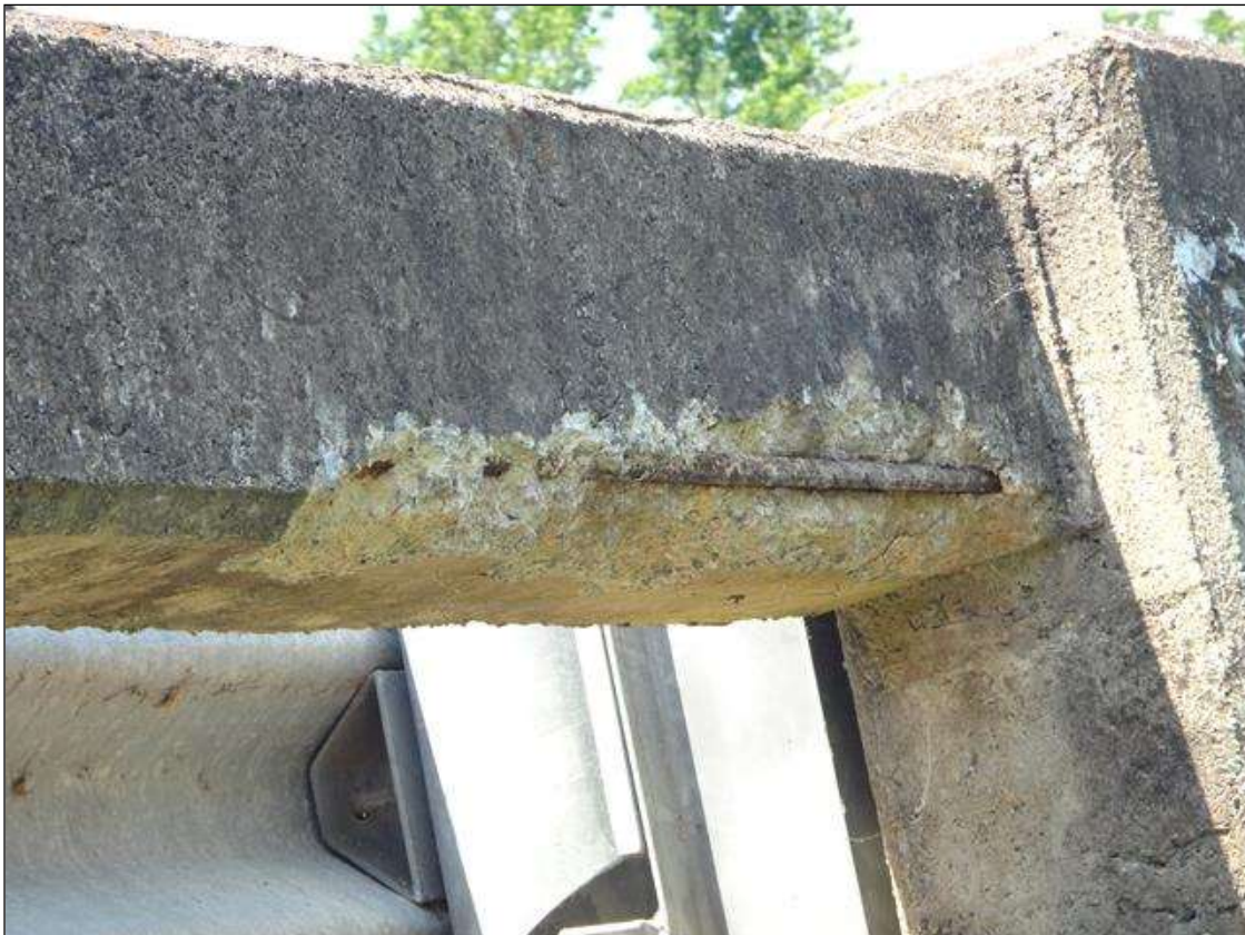
NORTH RAIL AT 16FT FROM END BENT 2, SPALL (3FT X 6IN X 2IN DEEP) WITH EXPOSED RUSTED REBAR
