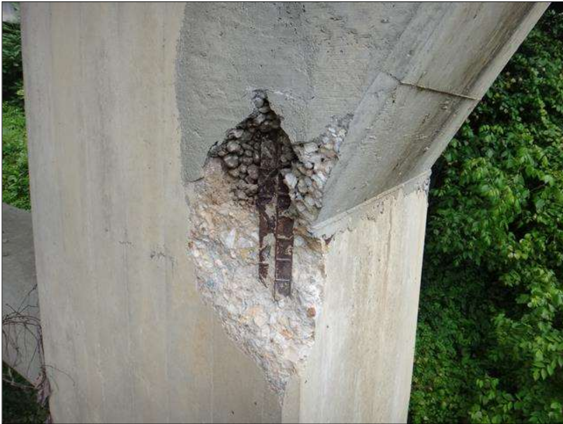
(PM) BENT 9 COLUMN 2 SOUTHWEST CORNER, SPALL (20IN X 12IN X 4IN DEEP) WITH EXPOSED RUSTED REBAR
