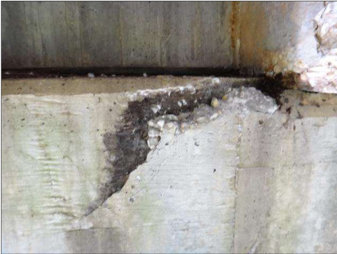
(PM) BENT 8 CAP EAST FACE BELOW BEAM 4, SPALL (2FT X 4IN X 2-1/2IN DEEP) WITH ADJACENT DELAMINATION
