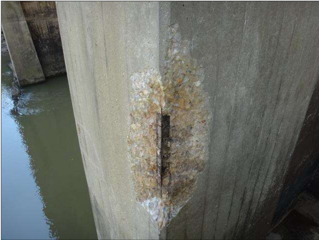
(PM) BENT 7 COLUMN 1 NORTHWEST CORNER AT 18FT FROM BOTTOM, SPALL (34IN X 9IN X 3IN DEEP) WITH EXPOSED RUSTED REBAR, SECTION LOSS (NO MEASURABLE LOSS)
