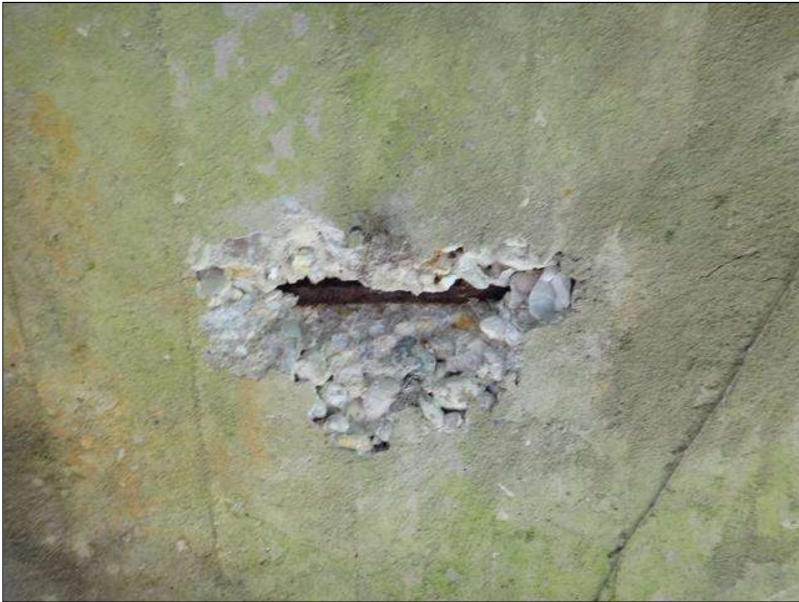
(PM) BENT 1 CAP UNDERSIDE BETWEEN COLUMNS 1 AND 2, SPALL (10IN X 7IN X 2IN DEEP) WITH EXPOSED RUSTED REBAR
