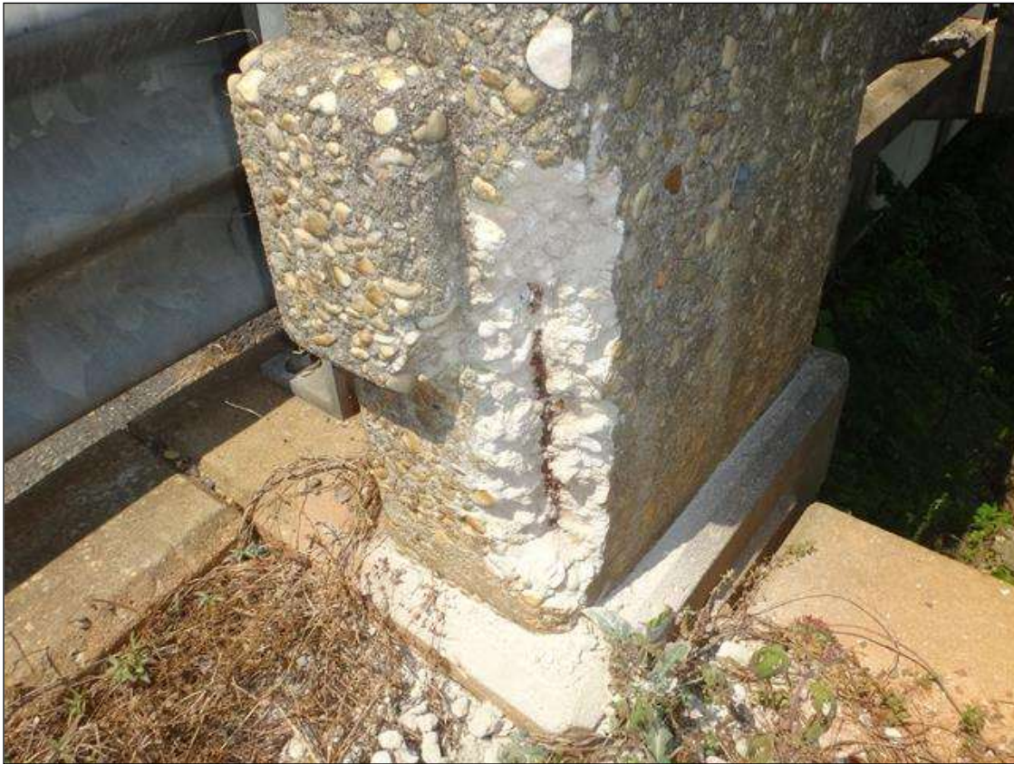
NORTH RAIL END POST AT END BENT 2, SPALL (18IN X 4IN X 2IN DEEP) WITH EXPOSED RUSTED REBAR
