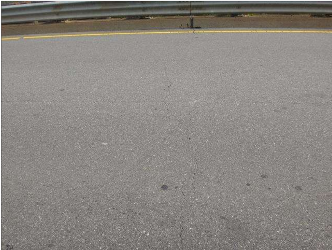
ASPHALT WEARING SURFACE OVER BENT 5, TRANSVERSE CRACK (FULL WIDTH X 1/8IN)
