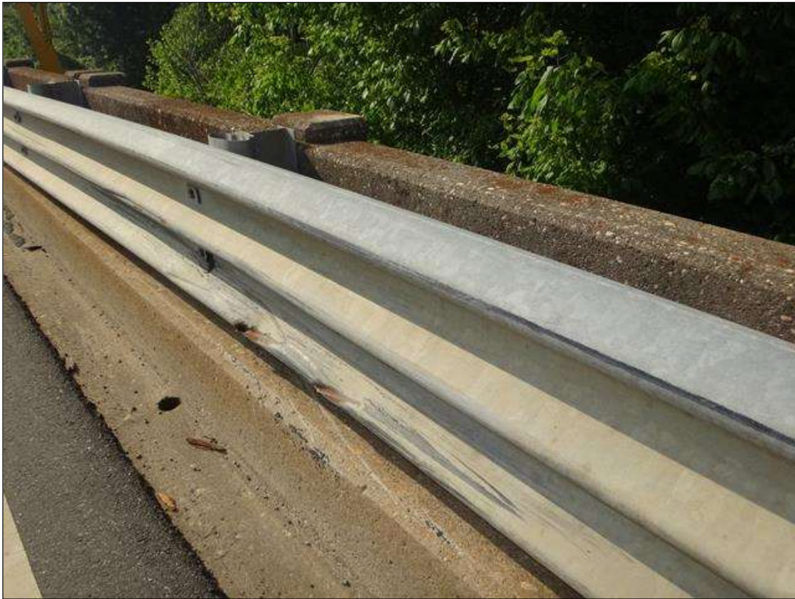
SPAN 1 SOUTH RAIL AT 25FT FROM END BENT 1, IMPACT DAMAGE (8FT)
