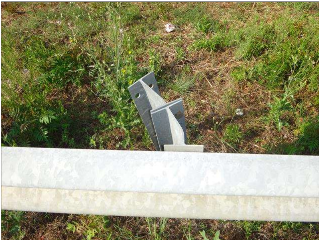
SOUTHWEST GUARDRAIL POST AT 100FT FROM END BENT 1, BENT/ROTATED (45 DEGREES)
