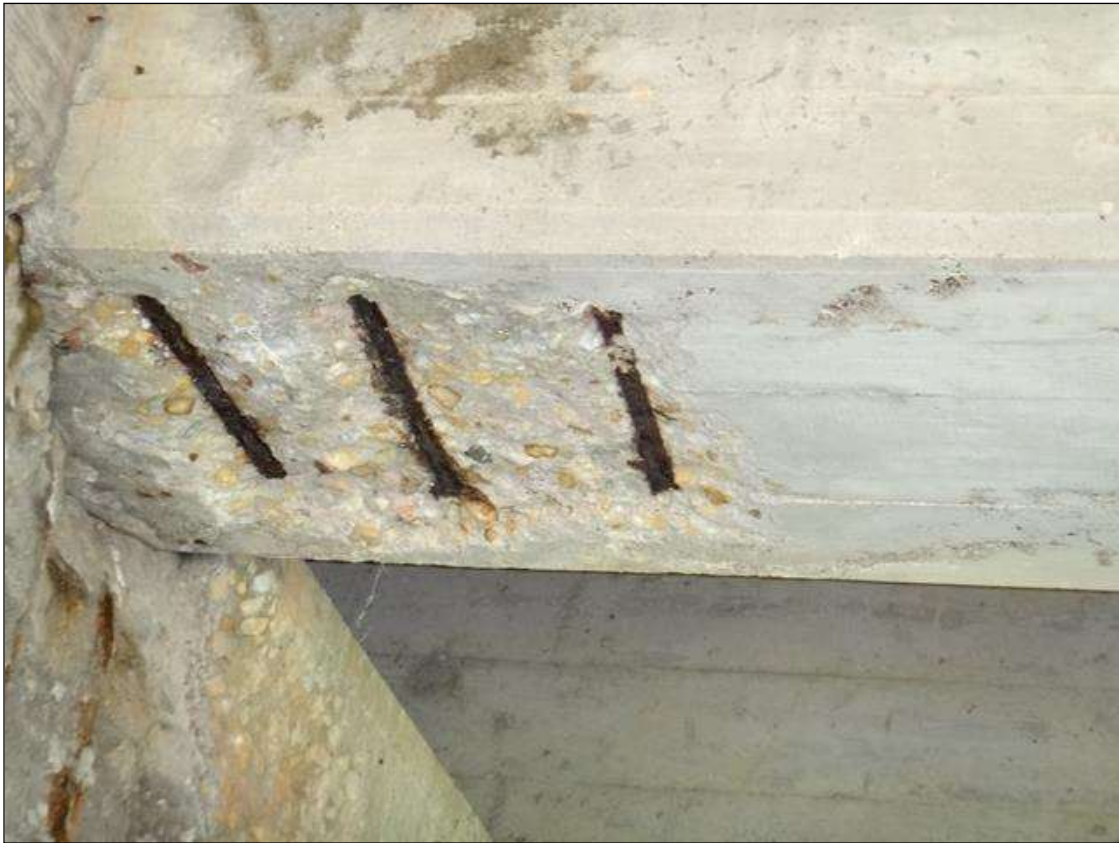
(PM) SPAN 1 BEAM 4 AT BENT 1, SPALL (18IN X 18IN X 2IN DEEP) WITH EXPOSED RUSTED REBAR, SECTION LOSS (NO MEASURABLE LOSS)
