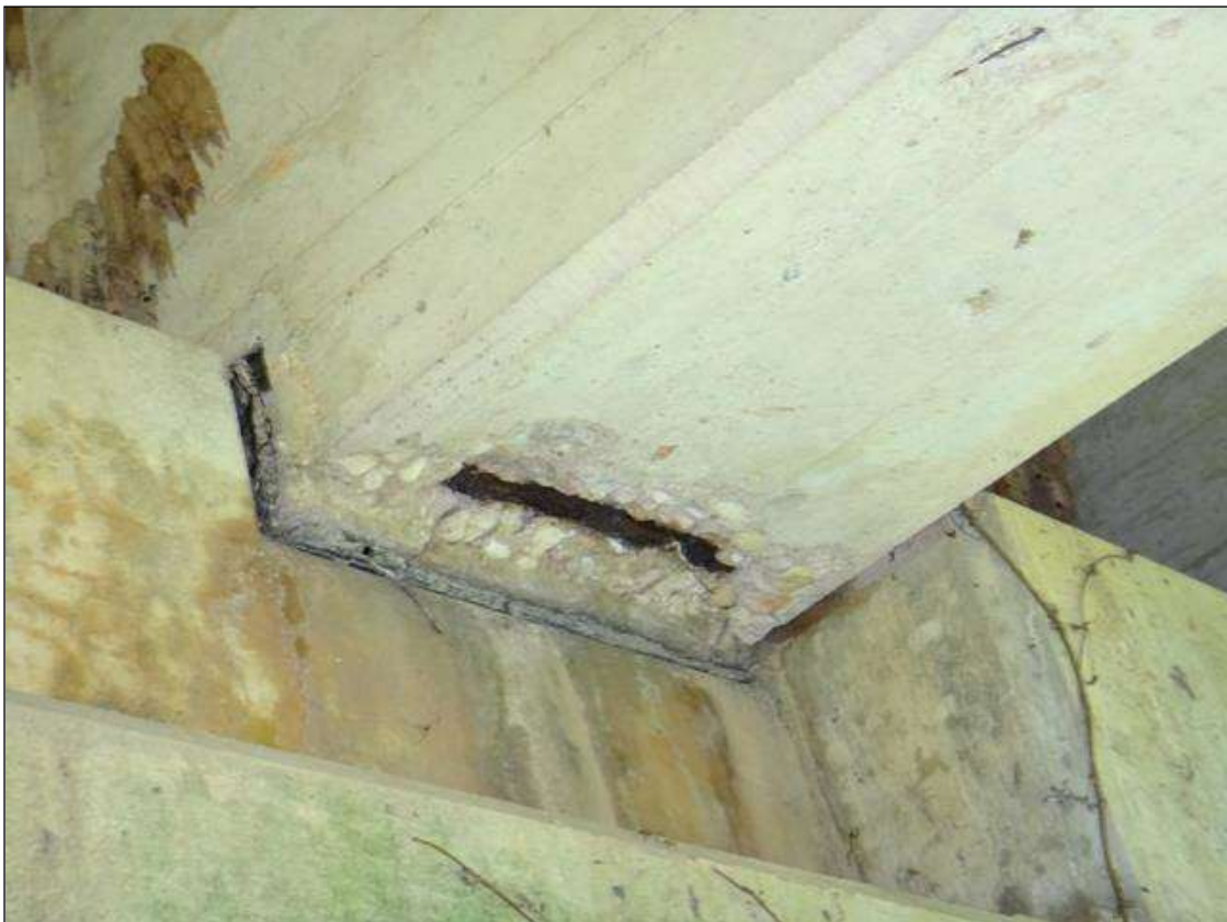
(PM) SPAN 10 BEAM 2 AT BENT 9, SPALL (18IN X 5IN X 2-1/2IN DEEP) WITH EXPOSED RUSTED REBAR
