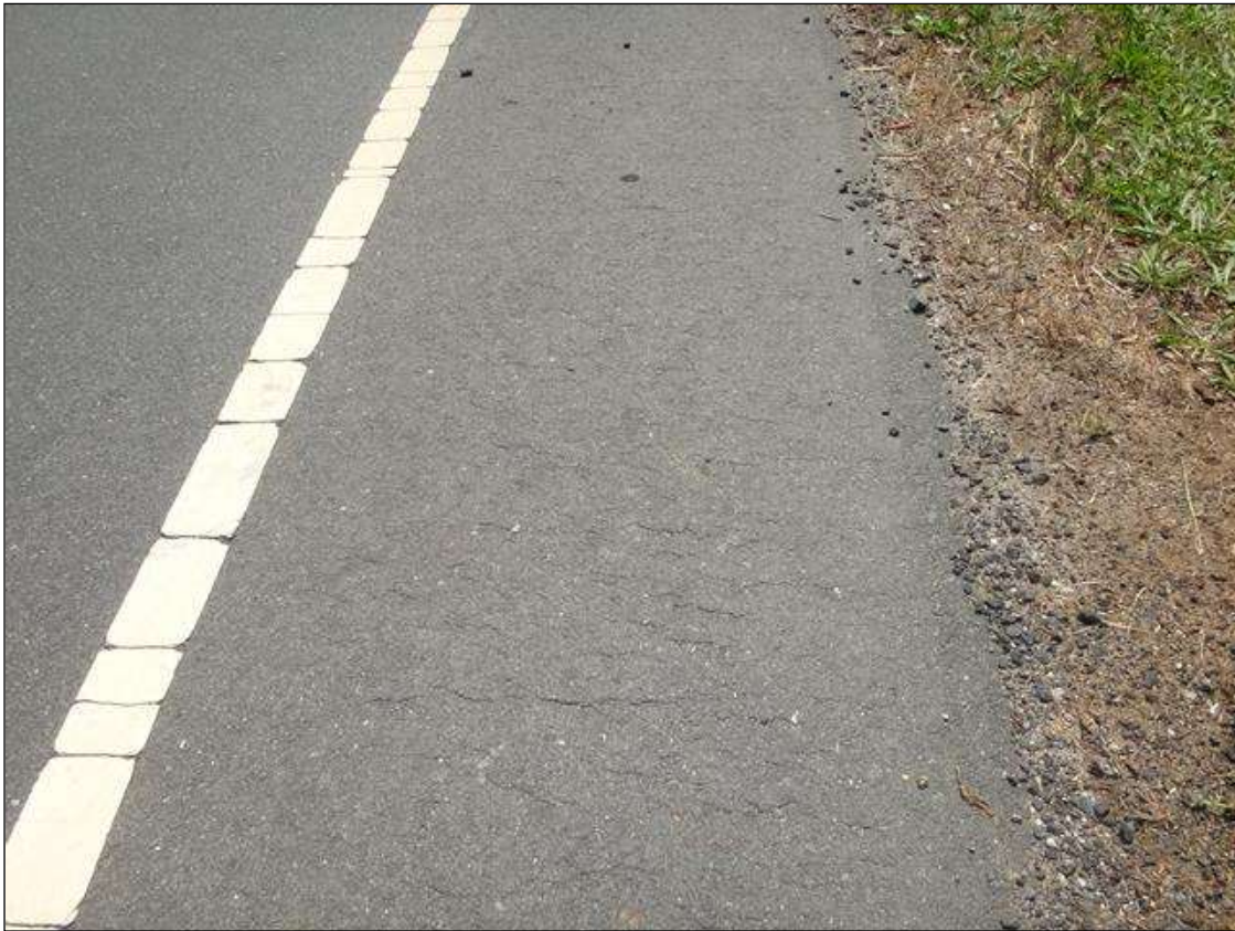
EAST APPROACH SOUTH SHOULDER ASPHALT WEARING SURFACE, ASPHALT RAVELING (25FT X 3FT)
