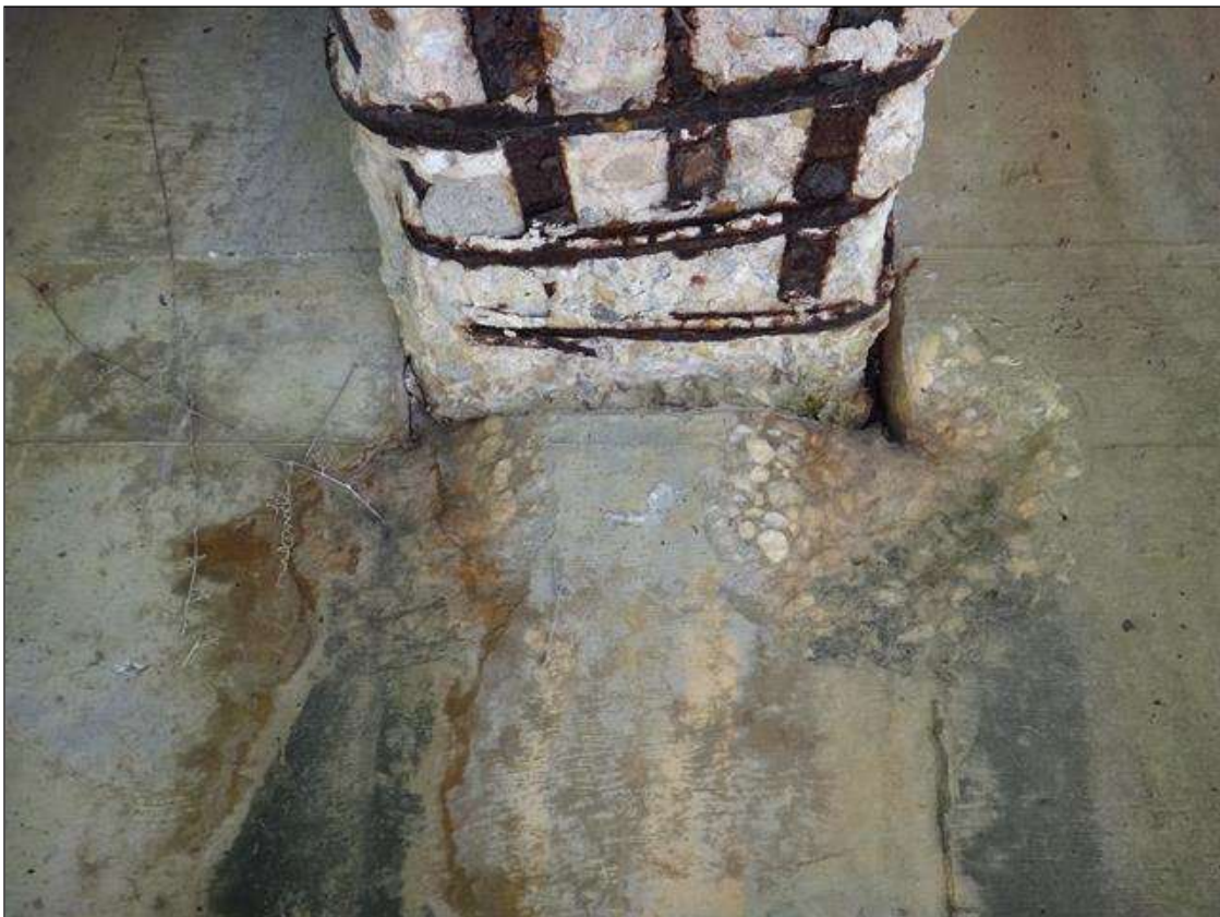
BENT 1 CAP EAST FACE BELOW BEAM 3, TWO (2) SPALLS (UP TO 14IN DIAMETER X 2IN DEEP)
