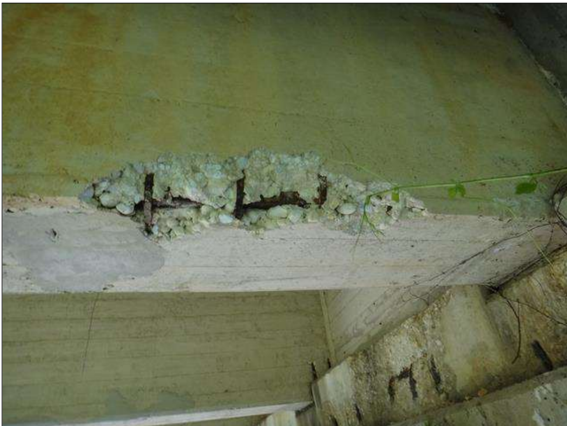
(PM) SPAN 4 BEAM 4 AT BENT 4, SPALL (2FT X 6IN X 4IN DEEP) WITH EXPOSED RUSTED REBAR
