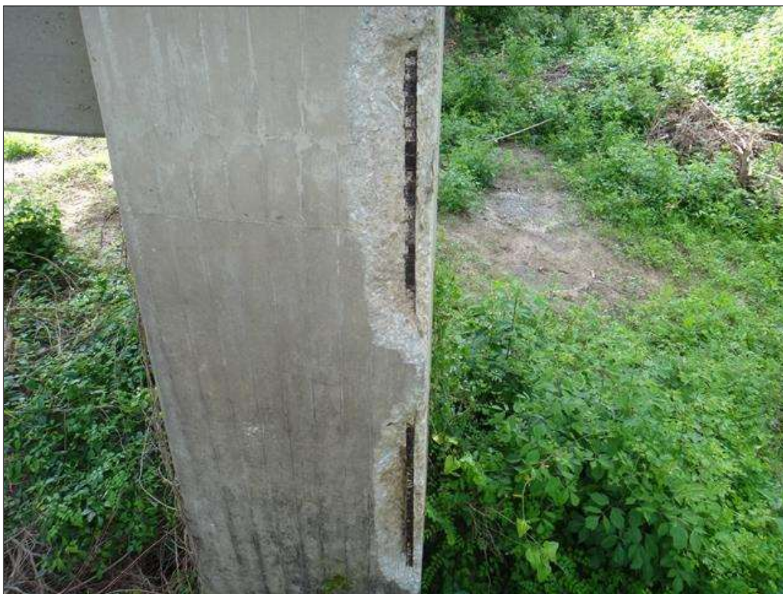
(PM) BENT 3 COLUMN 2 SOUTHWEST CORNER, TWO (2) SPALLS (UP TO 4FT X 15IN X 4IN DEEP) WITH EXPOSED RUSTED REBAR, SECTION LOSS (NO MEASURABLE LOSS)
