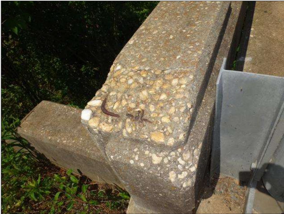
SOUTH RAIL END POST AT END BENT 2, SPALL (10IN X 8IN X 1IN DEEP) WITH EXPOSED RUSTED REBAR
