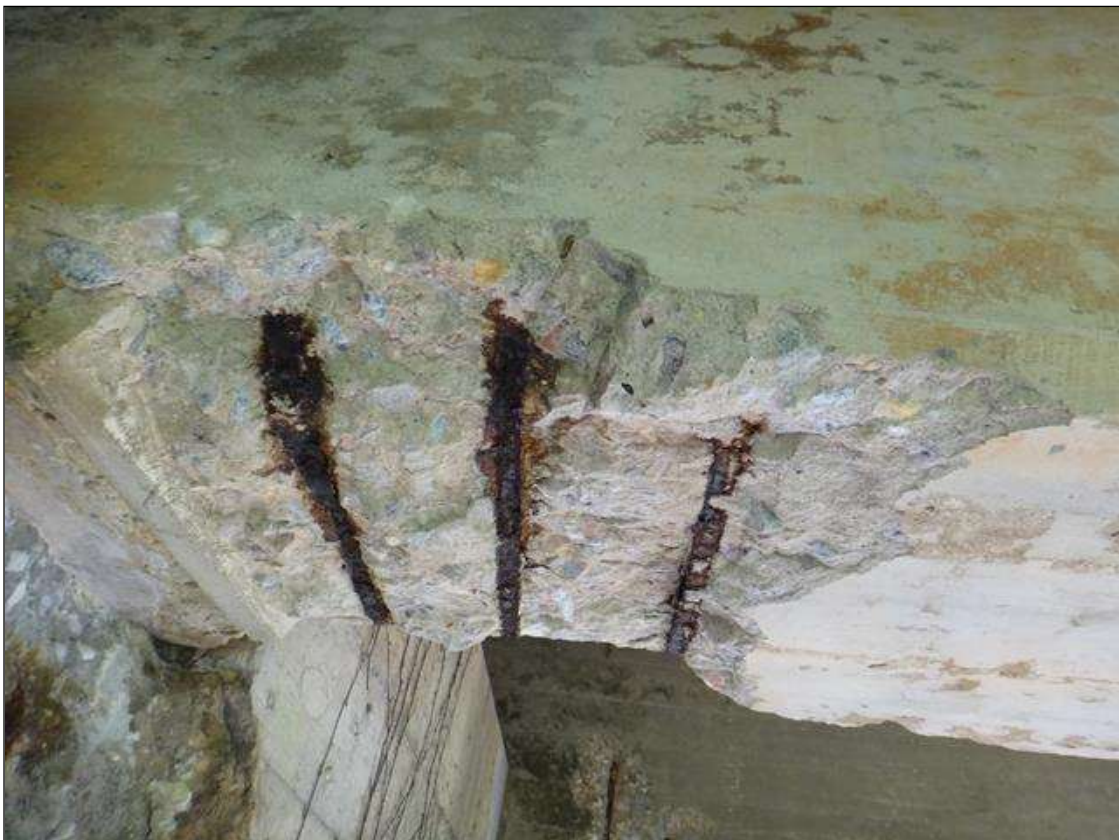
(PM) SPAN 2 BEAM 4 AT BENT 1, SPALL (2FT X 2FT X 2IN DEEP) WITH EXPOSED RUSTED REBAR AND SECTION LOSS ON REBAR
