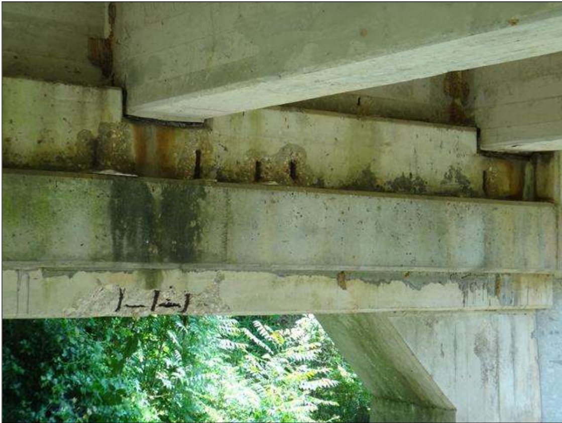
(PM) BENT 9 CAP WEST FACE, MULTIPLE SPALLS (UP TO 3-1/2FT X 12IN X 4IN DEEP) WITH EXPOSED RUSTED REBAR, SECTION LOSS (NO MEASURABLE LOSS)
