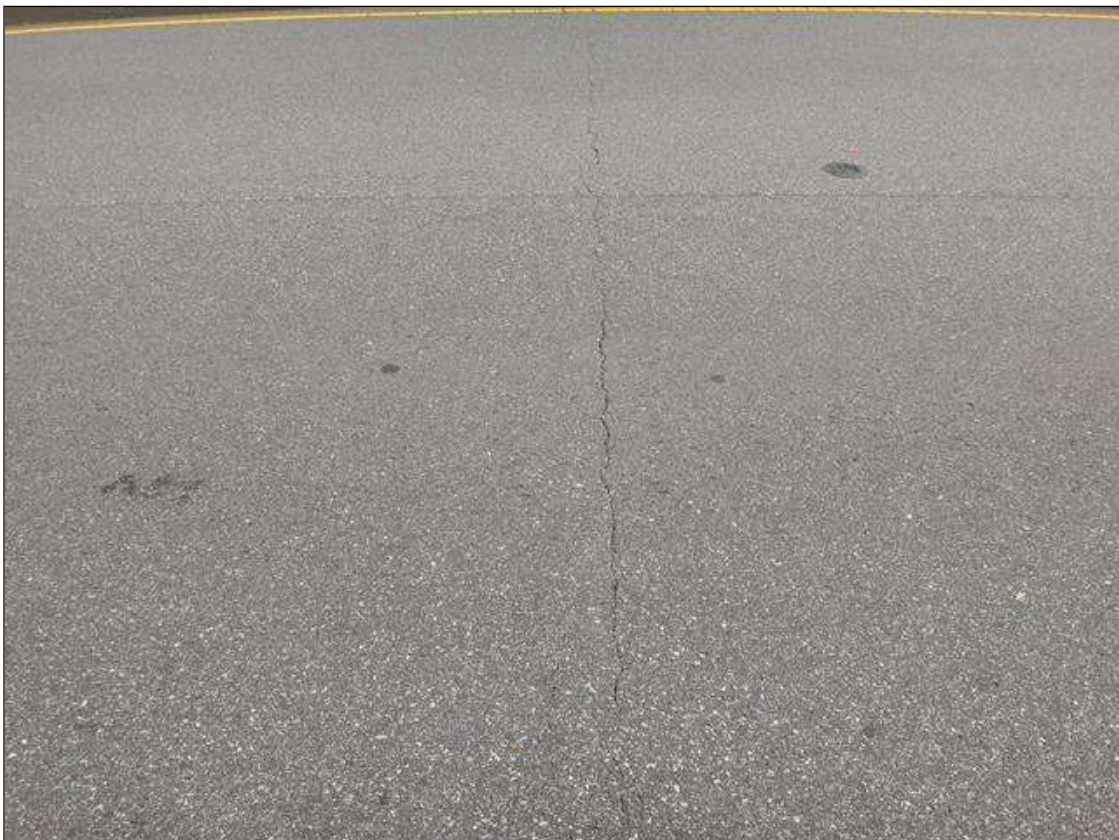
ASPHALT WEARING SURFACE OVER BENT 4, TRANSVERSE CRACK (FULL WIDTH X 1/8IN)
