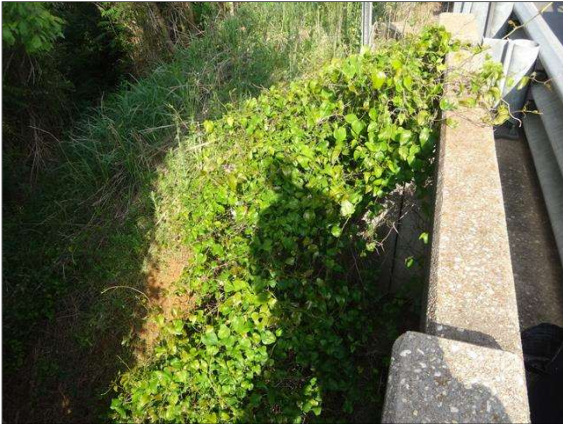
SOUTH RAIL AND SOUTHWEST EARWALL AT END BENT 1, VEGETATION GROWTH (15FT X 10FT X 3FT)
