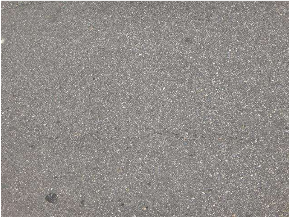
SPAN 7 ASPHALT WEARING SURFACE RIGHT LANE AT 3FT FROM BENT 6, LONGITUDINAL CRACK (4FT X 1/16IN)
