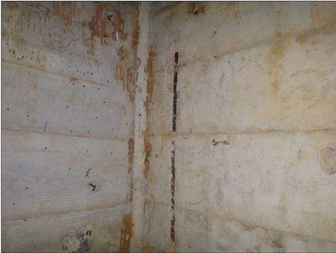
(PM) SPAN 10 BEAM 4 NORTH FACE AT END BENT 2, SPALL (2FT X 3IN X 1/2IN DEEP) WITH EXPOSED RUSTED REBAR
