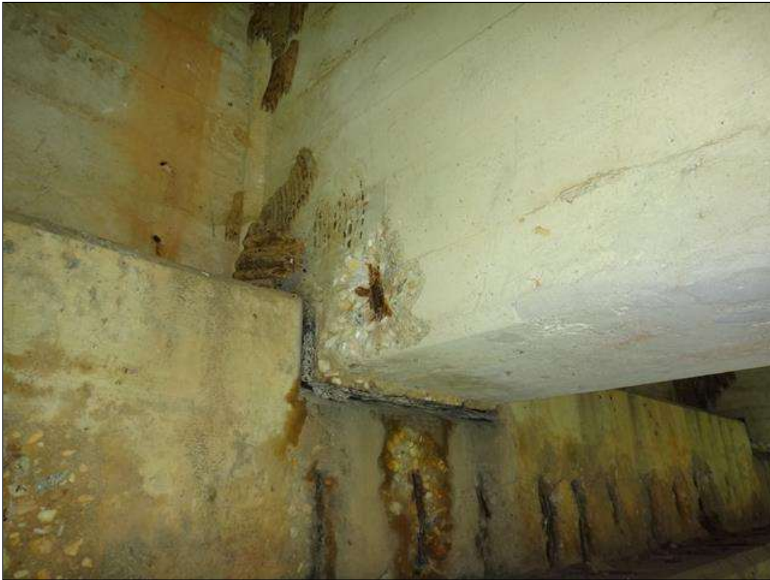
(PM) SPAN 10 BEAM 4 AT BENT 9, SPALL (6IN DIAMETER X 1-1/2IN DEEP) WITH EXPOSED RUSTED REBAR, SECTION LOSS (NO MEASURABLE LOSS)
