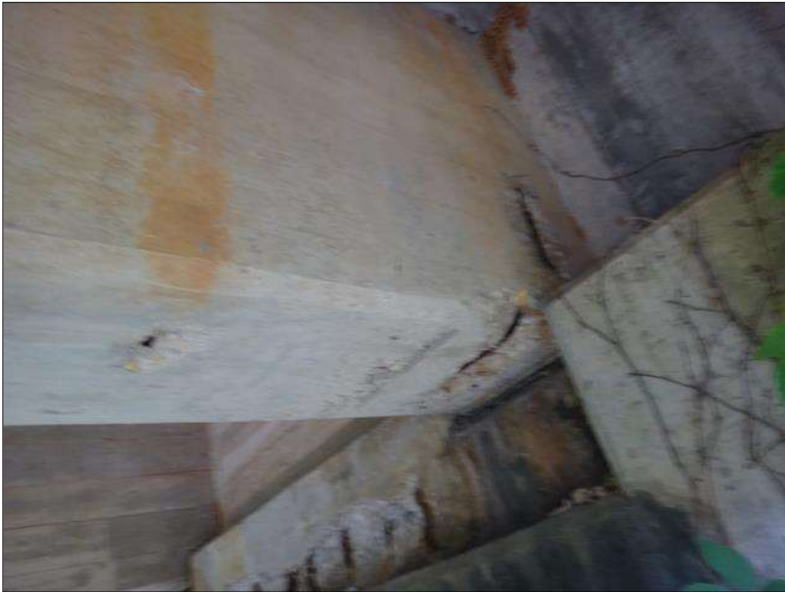
(PM) SPAN 3 BEAM 2 AT BENT 2, THREE (3) SPALLS (UP TO 16IN X 6IN X 2IN DEEP) WITH EXPOSED RUSTED REBAR
