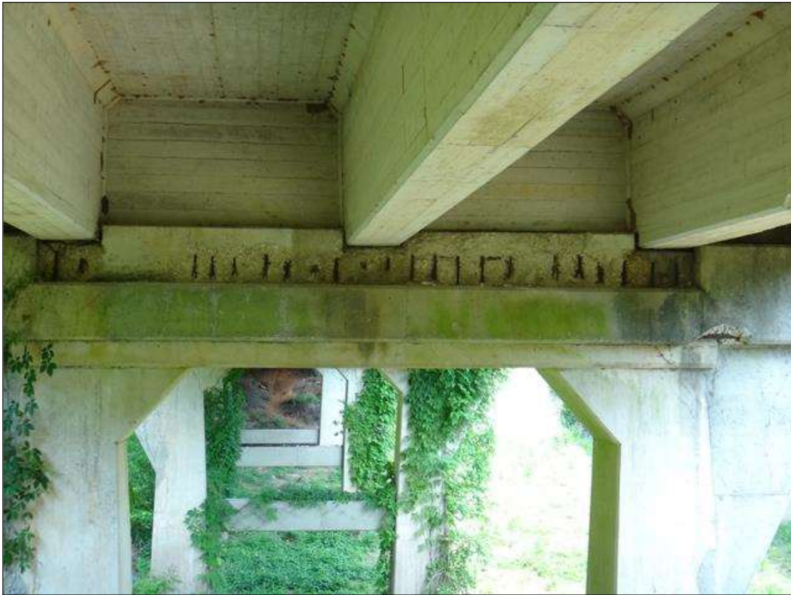
(PM) BENT 4 CAP EAST FACE, MULTIPLE SPALLS (UP TO 17FT X 20IN X 3IN DEEP) WITH EXPOSED RUSTED REBAR, SECTION LOSS (NO MEASURABLE LOSS)
