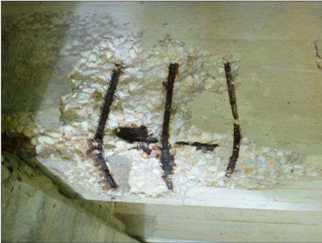
(PM) SPAN 9 BEAM 4 AT BENT 8, SPALL (2FT X 4IN X 2-1/2IN DEEP) WITH EXPOSED RUSTED REBAR, SECTION LOSS (NO MEASURABLE LOSS)
