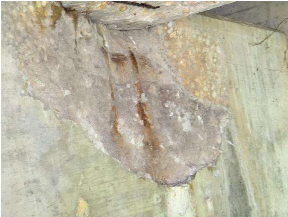
(PM) BENT 1 CAP WEST FACE BELOW BENT 4, SPALL (3FT X 20IN X 4IN DEEP) WITH EXPOSED RUSTED REBAR
