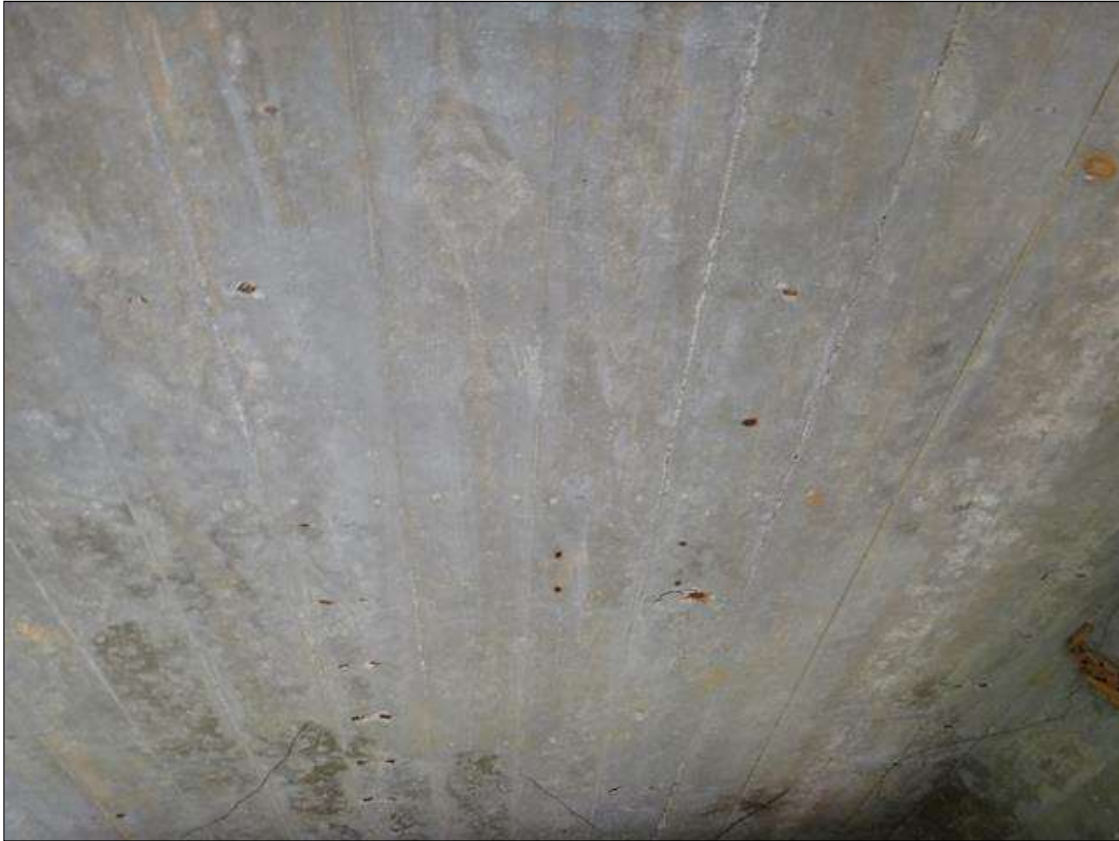
SPAN 2 UNDERSIDE OF DECK AT BAY 3, MULTIPLE POPOUTS/DELAMINATION (UP TO 1IN DIAMETER) WITH EXPOSED RUSTED REBAR (ALL BAYS SIMILAR)
