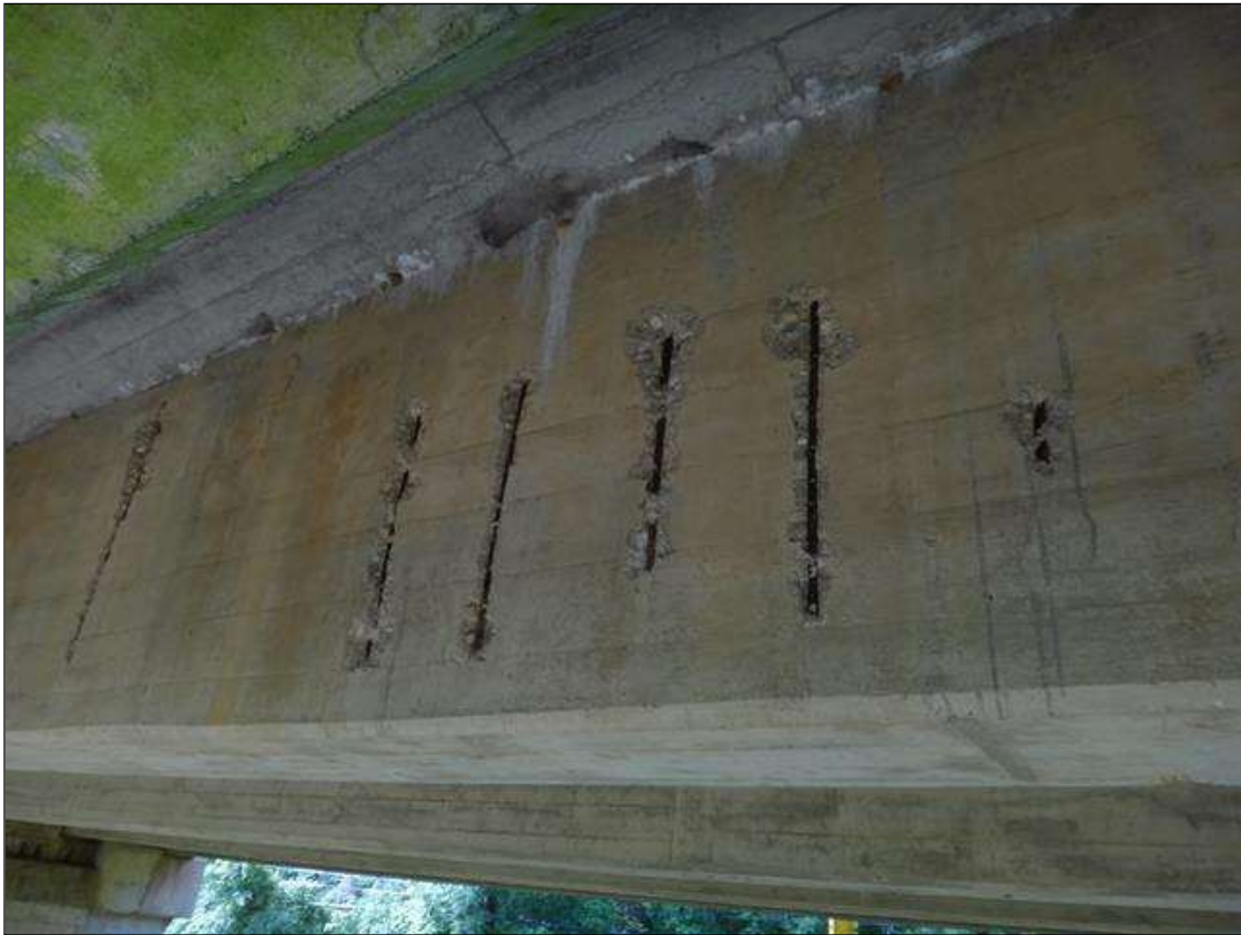
(PM) SPAN 3 BEAM 2 AT MIDSPAN, EIGHT (8) SPALLS AT STIRRUPS (UP TO 3FT X 5IN X 1IN DEEP) WITH EXPOSED RUSTED REBAR
