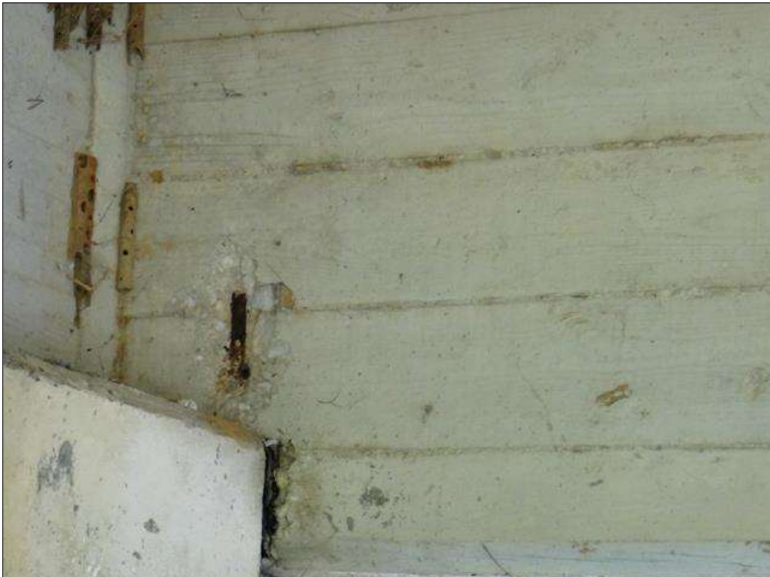
(PM) SPAN 7 BEAM 2 AT BENT 6, SPALL (6IN DIAMETER X 1IN DEEP) WITH EXPOSED RUSTED REBAR
