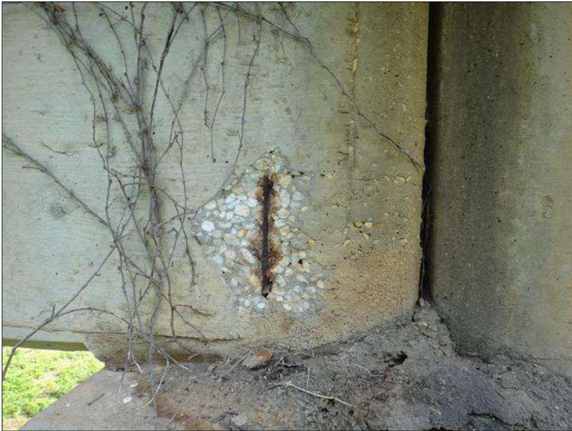
(PM) SPAN 3 BEAM 5 AT BENT 3, SPALL (10IN X 8IN X 1IN DEEP) WITH EXPOSED RUSTED REBAR
