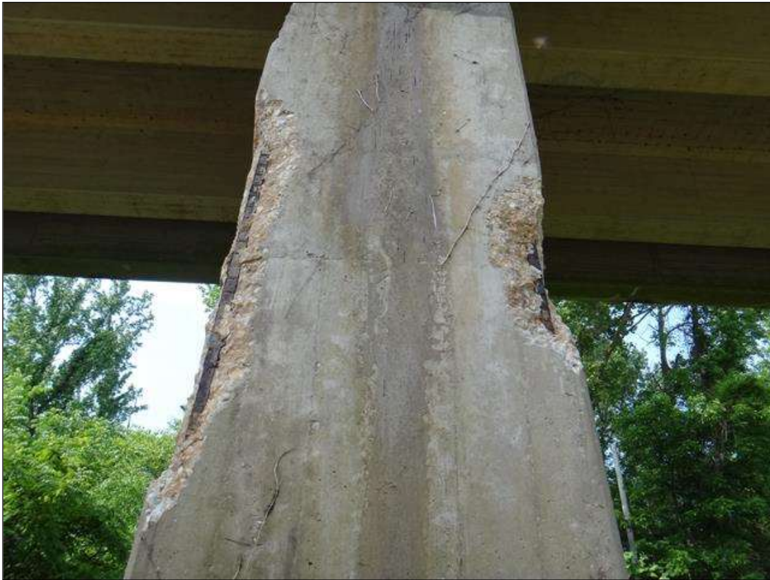
(PM) BENT 4 COLUMN 1 NORTH FACE, TWO (2) SPALLS (UP TO 5-1/2FT X 10IN X 3IN DEEP) WITH EXPOSED RUSTED REBAR, SECTION LOSS (NO MEASURABLE LOSS)
