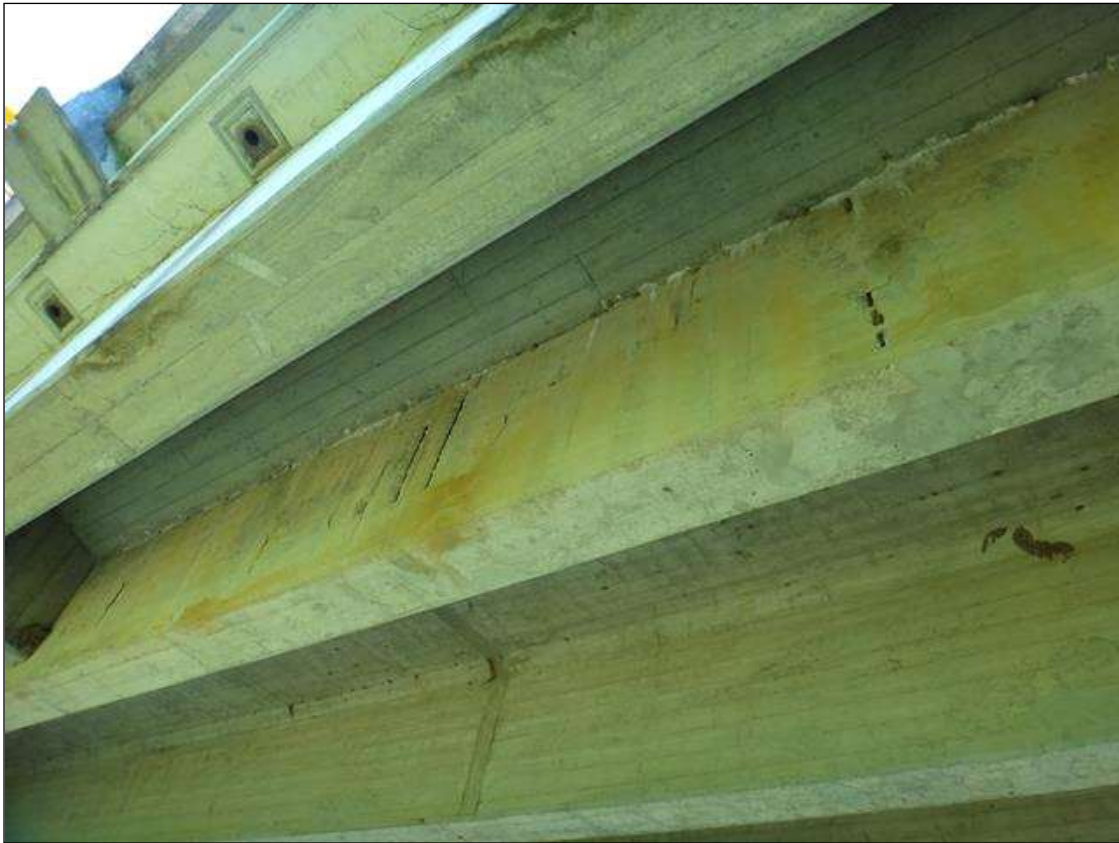
(PM) SPAN 6 BEAM 4 SOUTH FACE, MULTIPLE SPALLS (3FT X 4IN X 1IN) WITH EXPOSED RUSTED REBAR, MULTIPLE DELAMINATIONS (3FT X 3IN)
