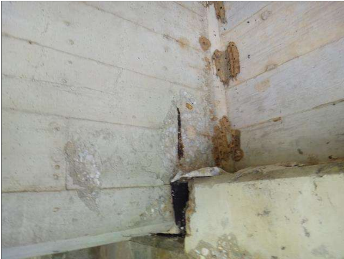
(PM) SPAN 7 BEAM 4 AT BENT 6, SPALL ON NORTH FACE (11IN X 6IN X 1IN DEEP) WITH EXPOSED RUSTED REBAR
