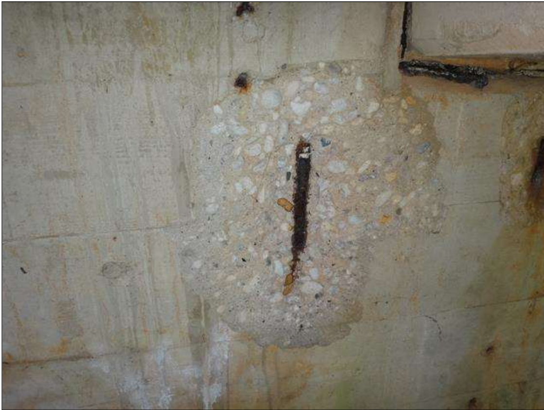
(PM) END BENT 2 CAP WEST FACE AT BEAM 3, SPALL (17IN X 15IN X 1IN DEEP) WITH EXPOSED RUSTED REBAR
