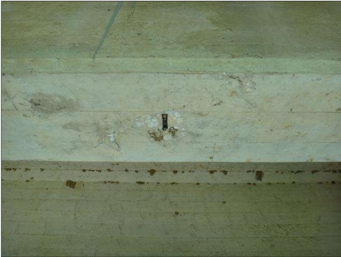
(PM) SPAN 8 BEAM 2 AT 8FT FROM BENT 7, SPALL (6IN DIAMETER X 1IN DEEP) WITH EXPOSED RUSTED REBAR AND ADJACENT DELAMINATION
