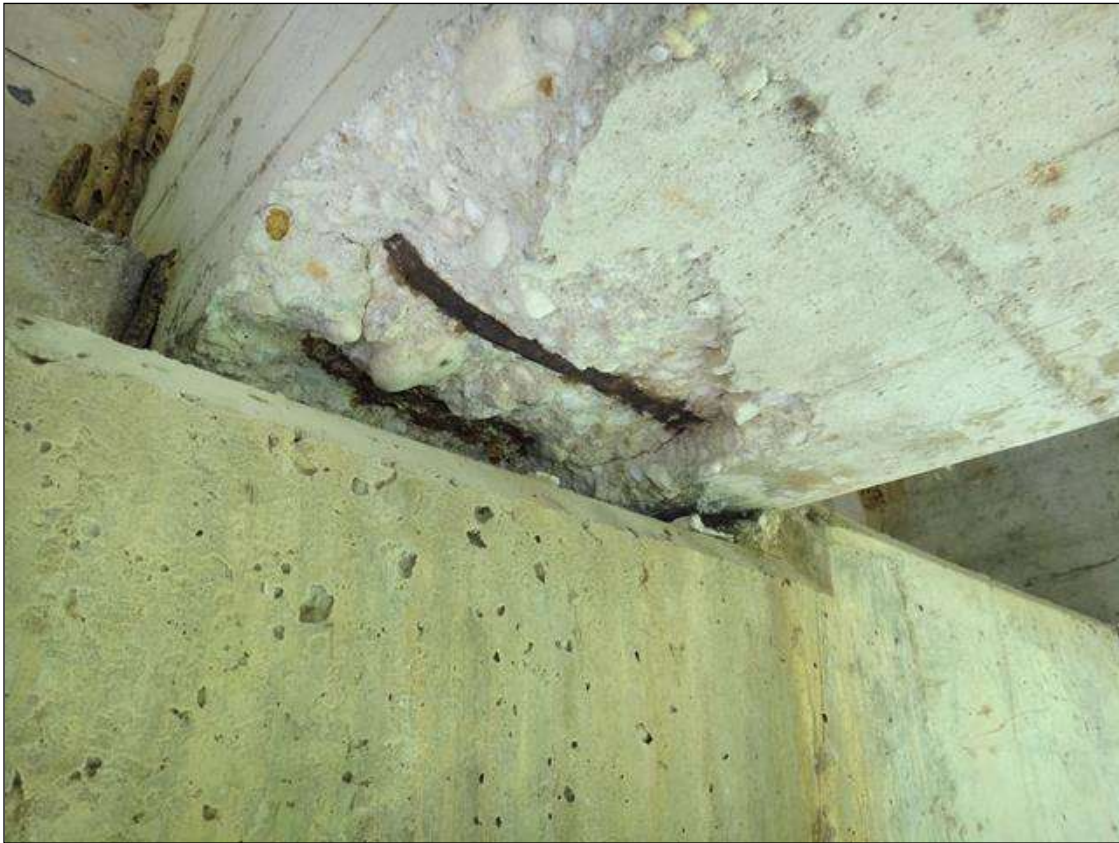
(PM) SPAN 7 BEAM 4 AT BENT 7, SPALL (16IN X 16IN X 2IN DEEP) WITH EXPOSED RUSTED REBAR AND ADJACENT DELAMINATION
