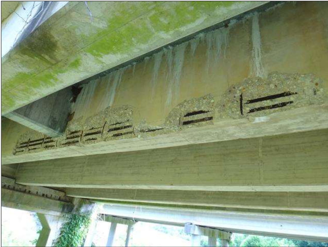
(PM) SPAN 3 BEAM 4 SOUTH FACE AT MIDSPAN, SPALL (18FT X 18IN X 2-1/2IN) WITH EXPOSED RUSTED REBAR, SECTION LOSS, DELAMINATION WITH TRANSVERSE CRACKS
