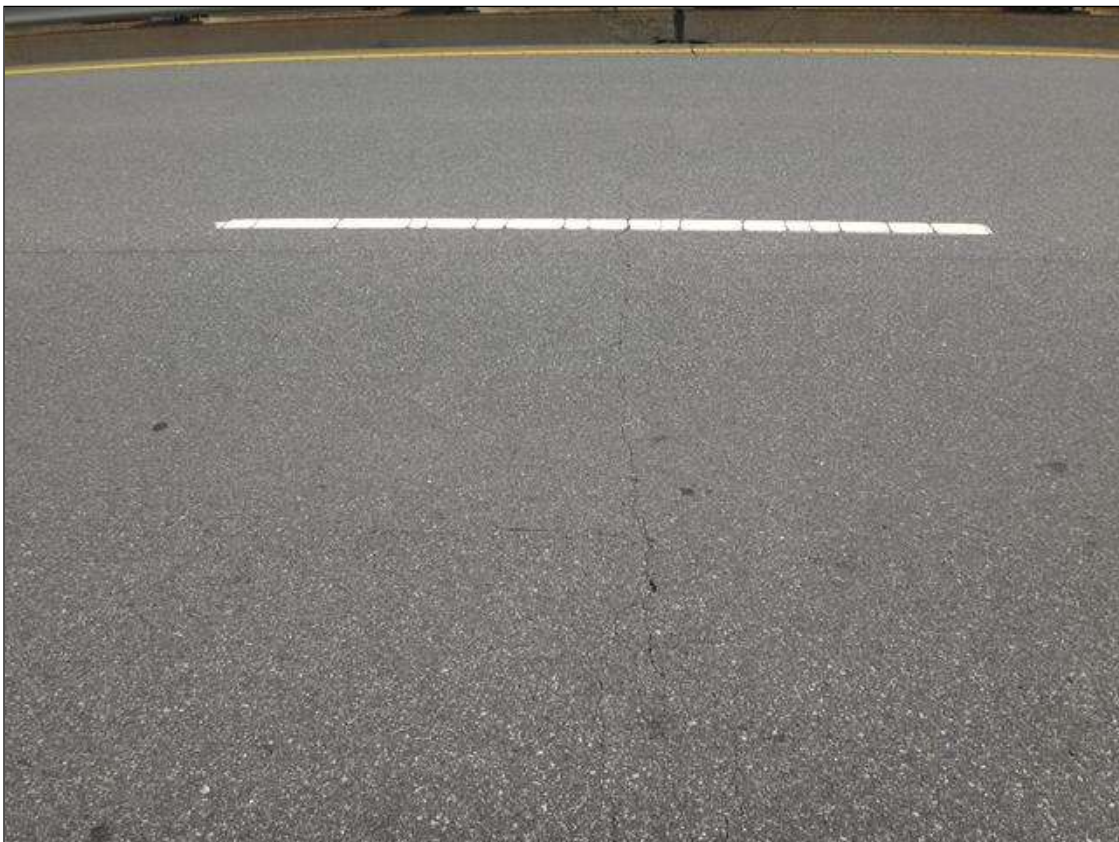
ASPHALT WEARING SURFACE OVER BENT 9, TRANSVERSE CRACK (FULL WIDTH X 1/8IN)
