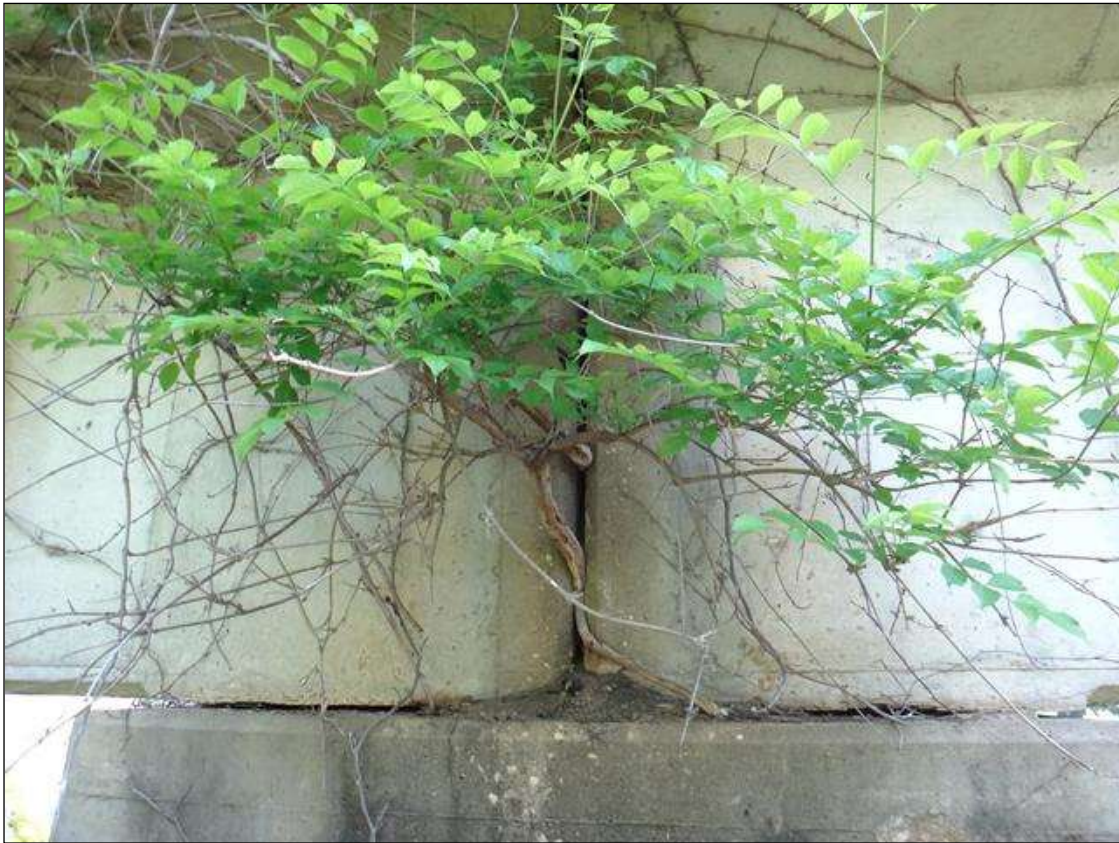
BENT 1 CAP SOUTH FACE, VEGETATION GROWTH (1CF) WITH DEBRIS ACCUMULATION (1CF)
