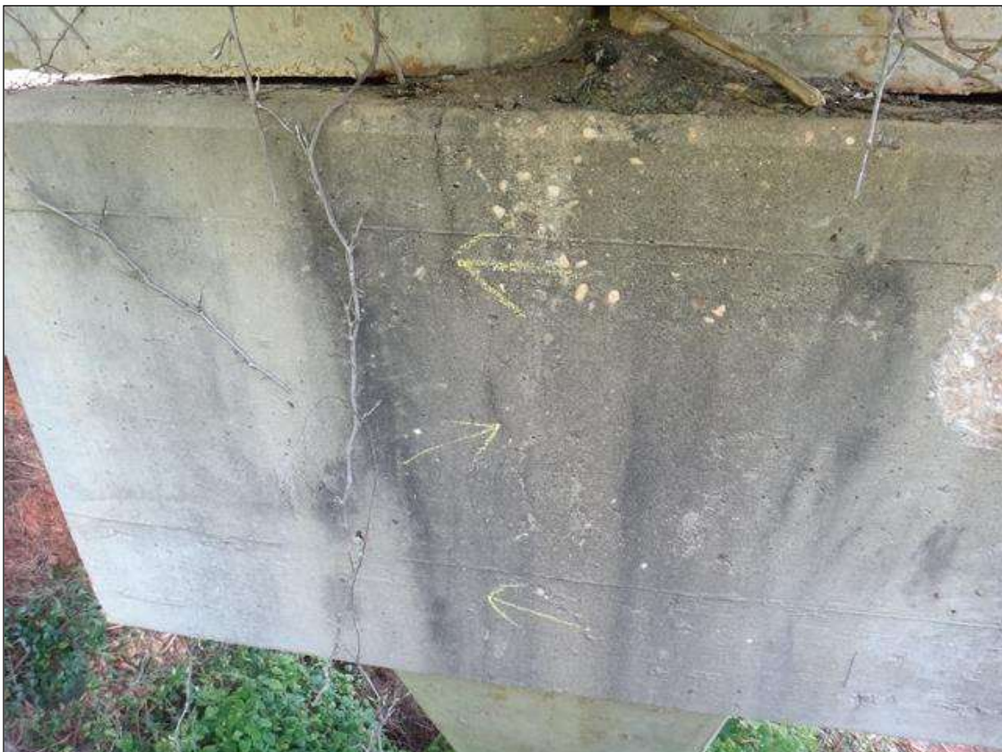
BENT 1 CAP SOUTH FACE, VERTICAL CRACK (FULL HEIGHT X HAIRLINE)
