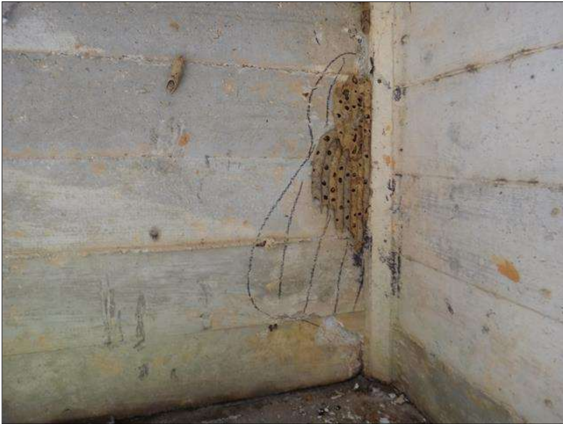
SPAN 8 BENT 8 BAY 3 BACKWALL AT BEAM 3, DELAMINATION (20IN X 9IN)
