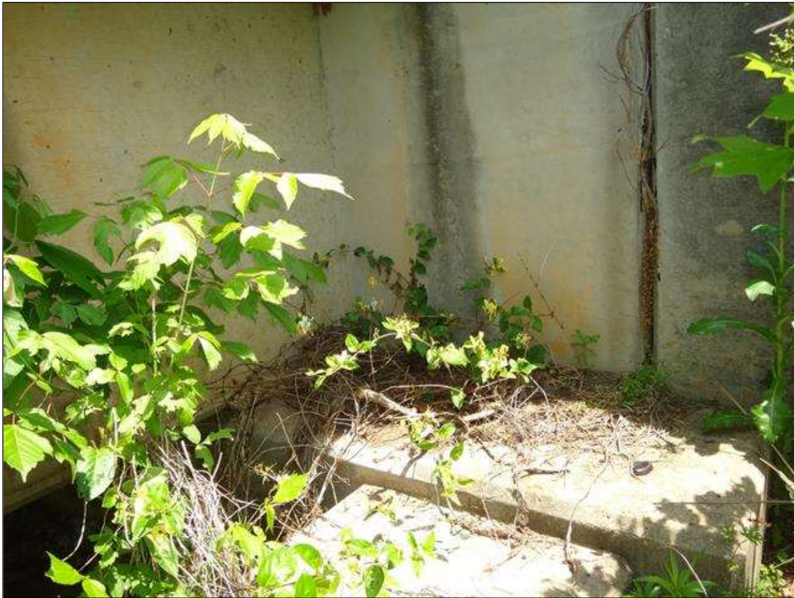
END BENT 2 CAP AT SOUTH END, DEBRIS ACCUMULATION WITH VEGETATION GROWTH (4FT X 2FT X 1FT)
