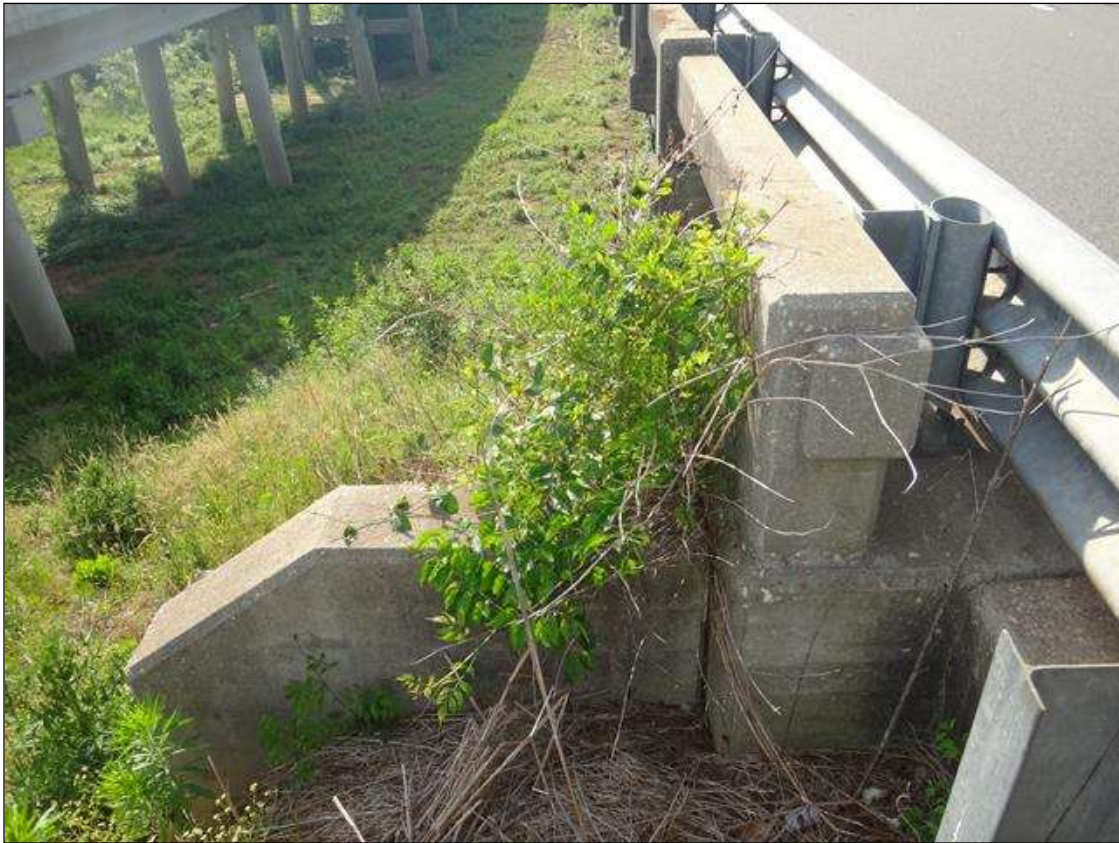
NORTH RAIL AND NORTHWEST EARWALL AT END BENT 1, VEGETATION GROWTH (5FT X 3FT X 5FT)
