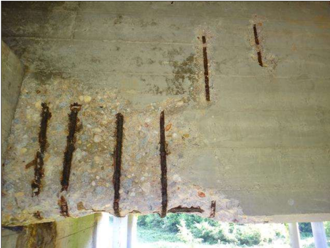
(PM) SPAN 2 BEAM 2 AT BENT 1, THREE (3) SPALLS (UP TO 36IN X 20IN X 2IN DEEP) WITH EXPOSED RUSTED REBAR, SECTION LOSS ON SECONDARY (UP TO 50%)
