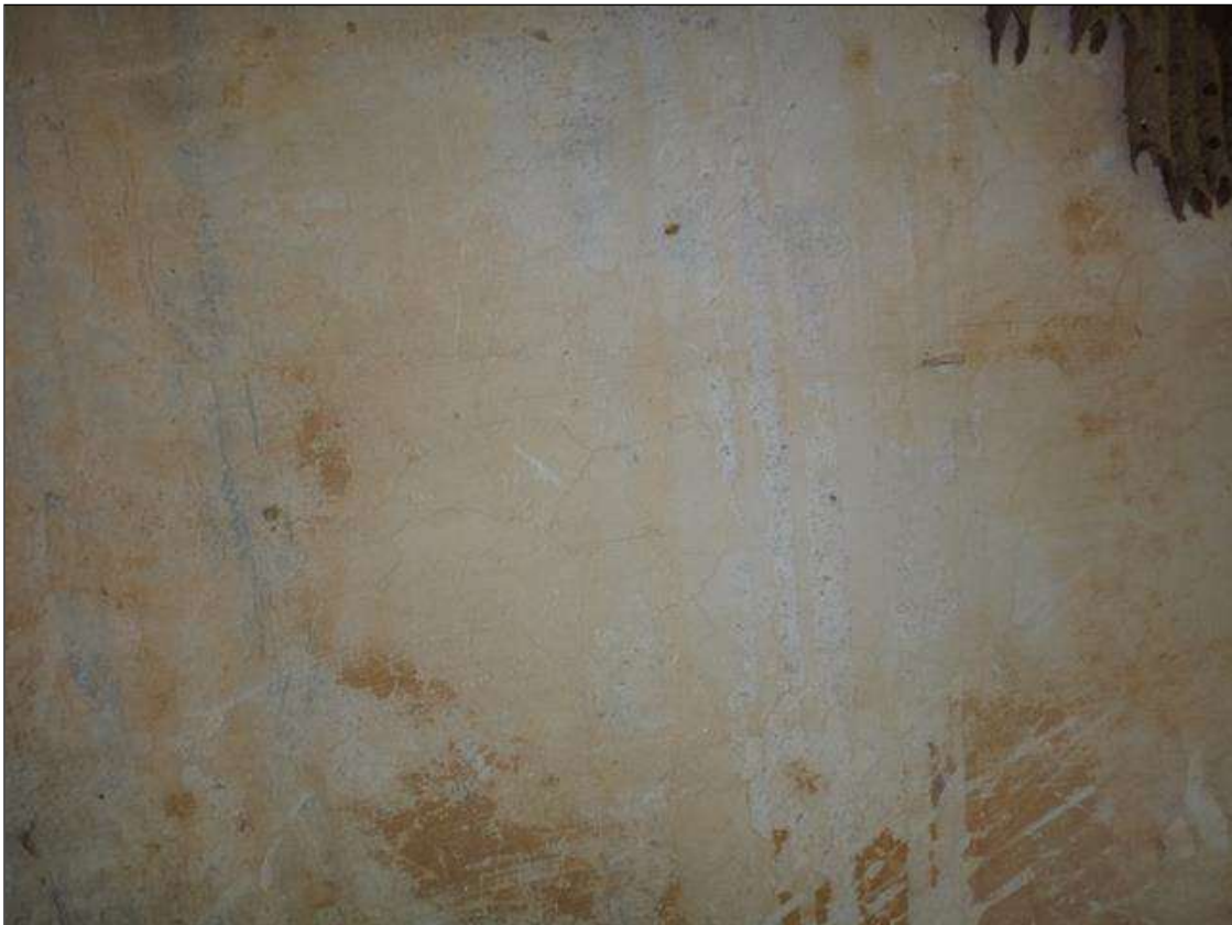
SPAN 10 BEAM 2 NORTH FACE AT END BENT 2, MAP CRACKING (3FT X 2FT X HAIRLINE)
