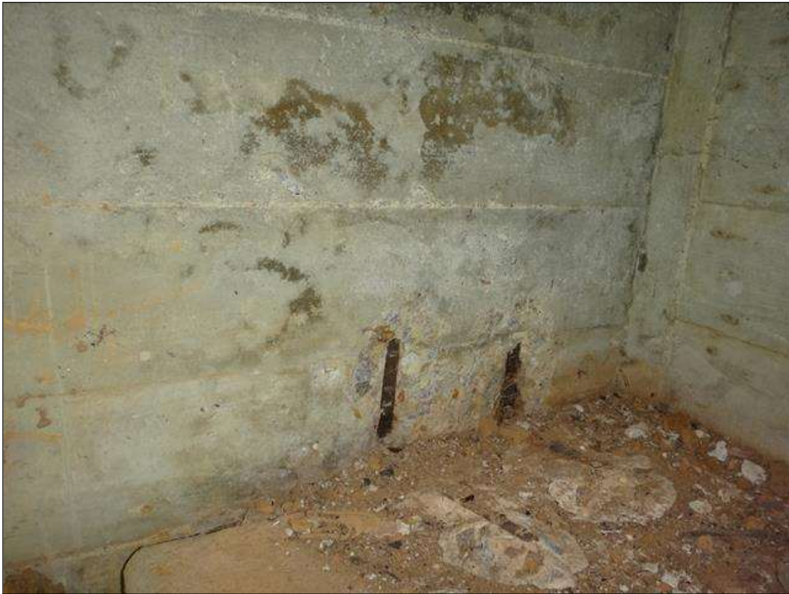
(PM) SPAN 1 BEAM 4 NORTH FACE AT END BENT 1, TWO (2) SPALLS (6IN X 4IN X 1IN DEEP) WITH EXPOSED RUSTED REBAR
