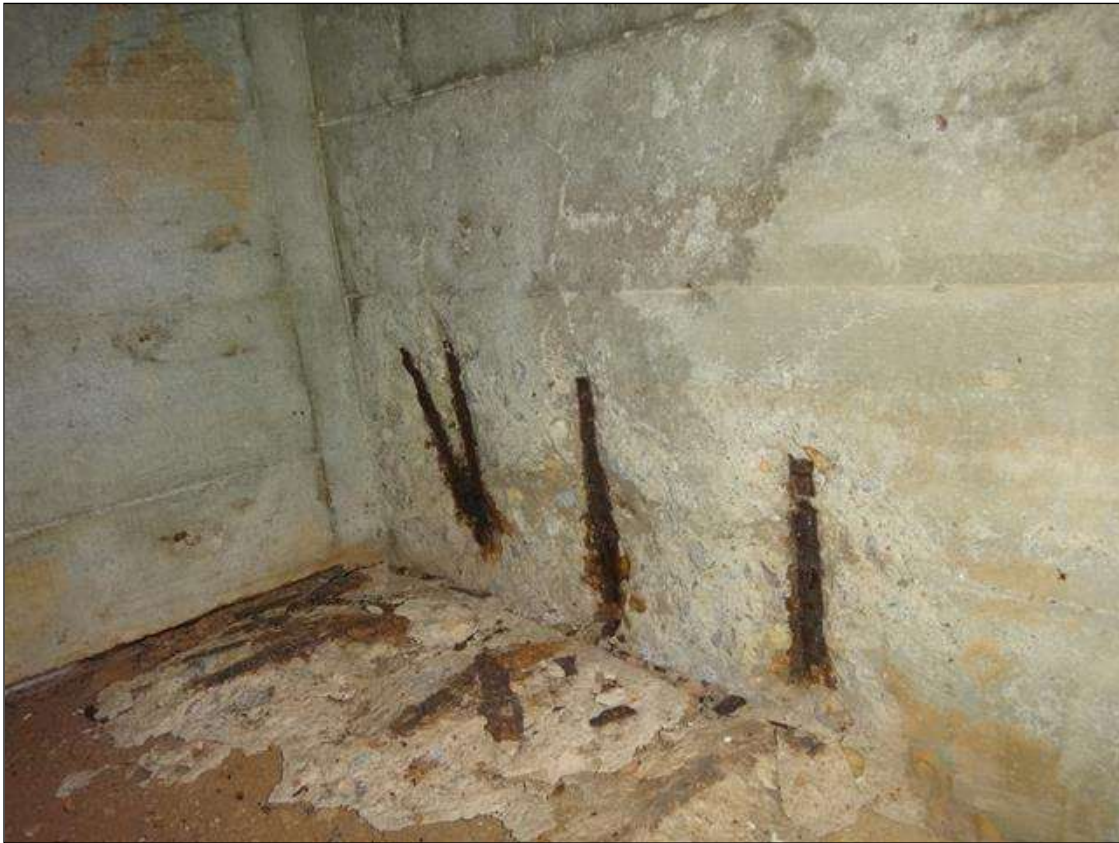
(PM) SPAN 1 BEAM 2 SOUTH FACE AT END BENT 1, THREE (3) SPALLS (UP TO 8IN X 6IN X 1IN DEEP) WITH EXPOSED RUSTED REBAR
