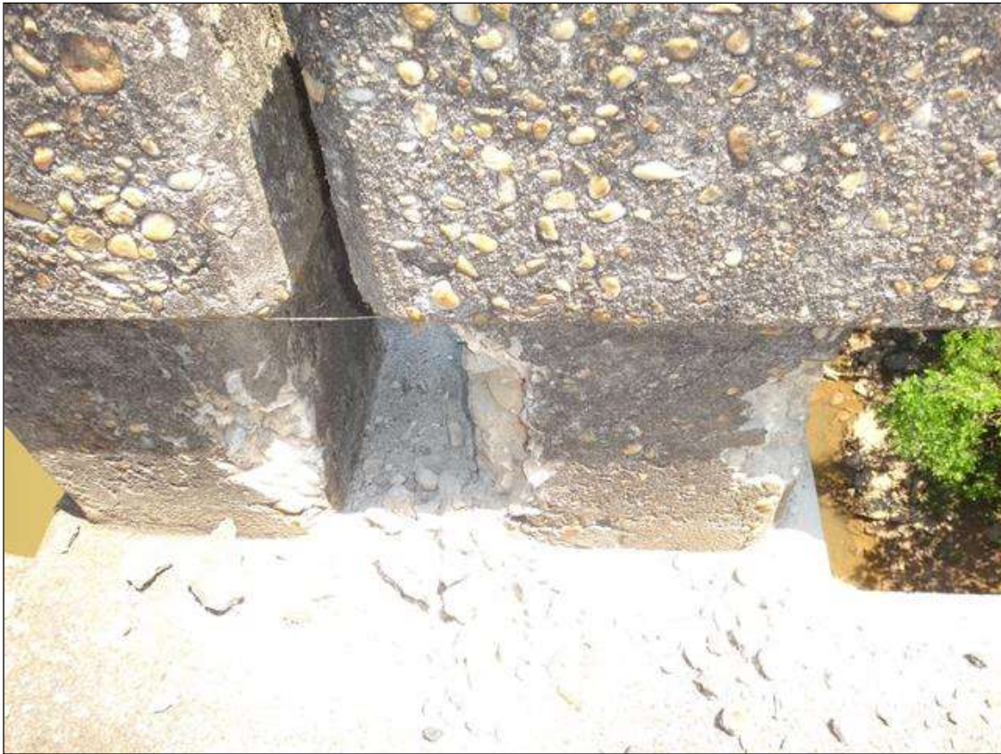
SPAN 9 NORTH RAIL POST NEAR MIDSPAN, THREE (3) SPALLS (UP TO 10IN X 5IN X 1-1/2IN DEEP) WITH EXPOSED RUSTED REBAR
