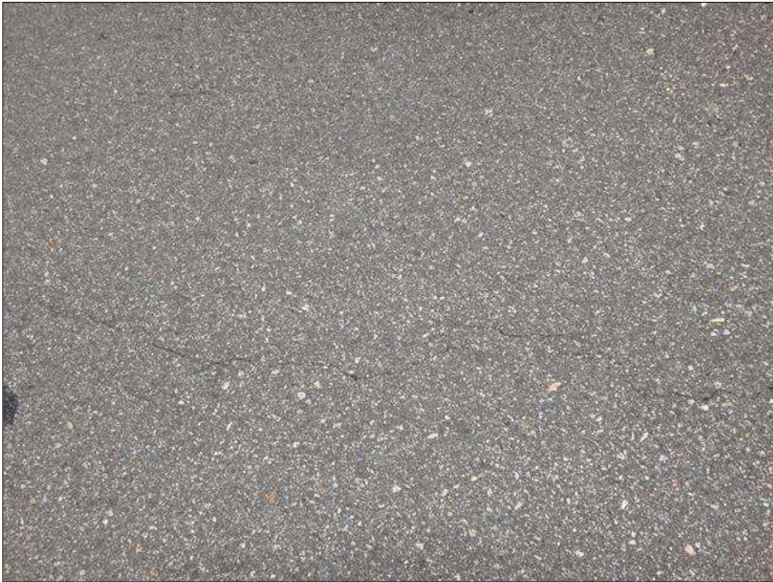
WEST APPROACH ASPHALT WEARING SURFACE AT END BENT 1, LONGITUDINAL CRACK (4FT X 1/16IN)
