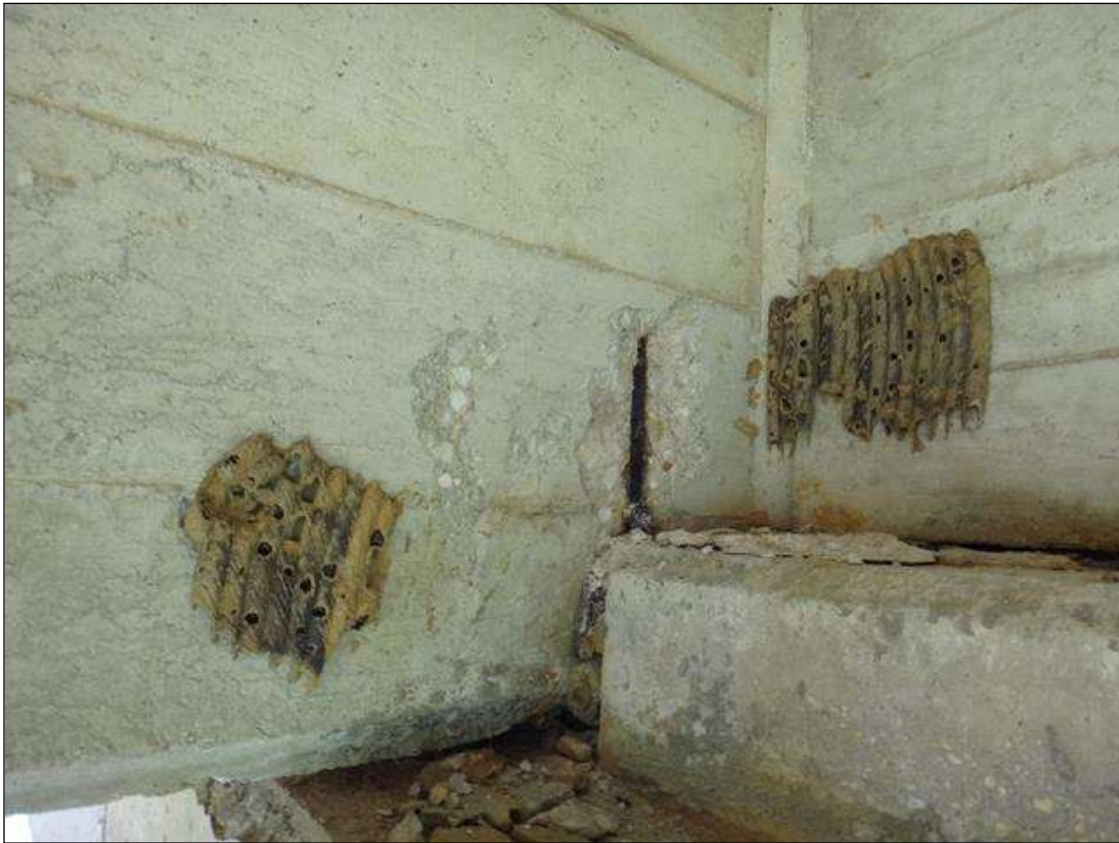
(PM) SPAN 7 BEAM 3 AT BENT 7, SPALL (10IN X 5IN X 1IN DEEP) WITH EXPOSED RUSTED REBAR AND ADJACENT DELAMINATION
