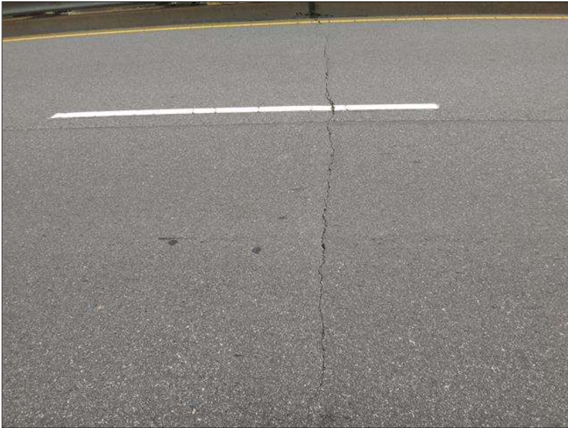
ASPHALT WEARING SURFACE OVER BENT 3, TRANSVERSE CRACK (FULL WIDTH X UP TO 1/4IN)
