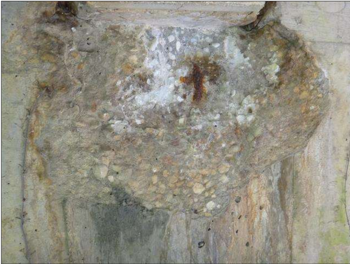
(PM) BENT 1 CAP EAST FACE BELOW BEAM 4, SPALL (18IN X 30IN X 3-1/2IN DEEP) WITH EXPOSED RUSTED REBAR
