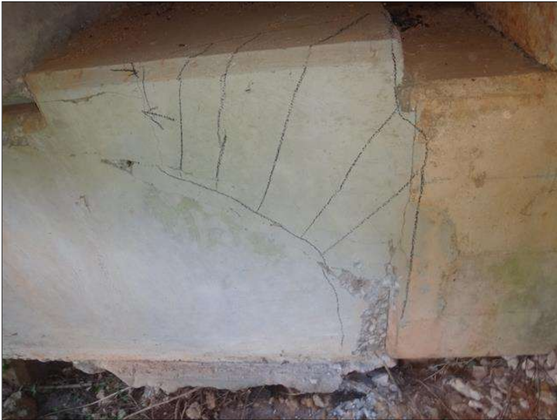
END BENT 2 BAY 1 WEST FACE AND TOP OF CAP, SPALL (15IN X 7IN X 1IN DEEP) WITH DELAMINATION (3FT X 2FT)
