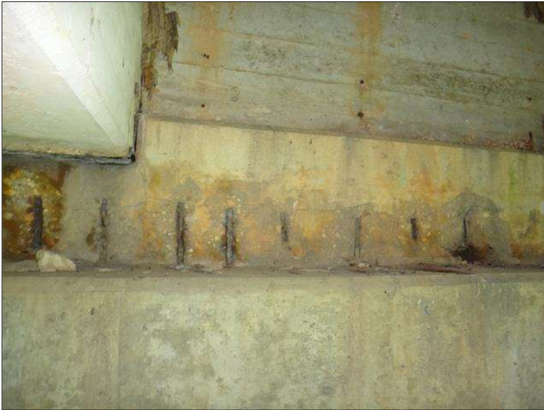
(PM) BENT 9 CAP EAST FACE, MULTIPLE SPALLS (UP TO 15FT X 13IN X 1-1/2IN DEEP) WITH EXPOSED RUSTED REBAR, SECTION LOSS (NO MEASURABLE LOSS)
