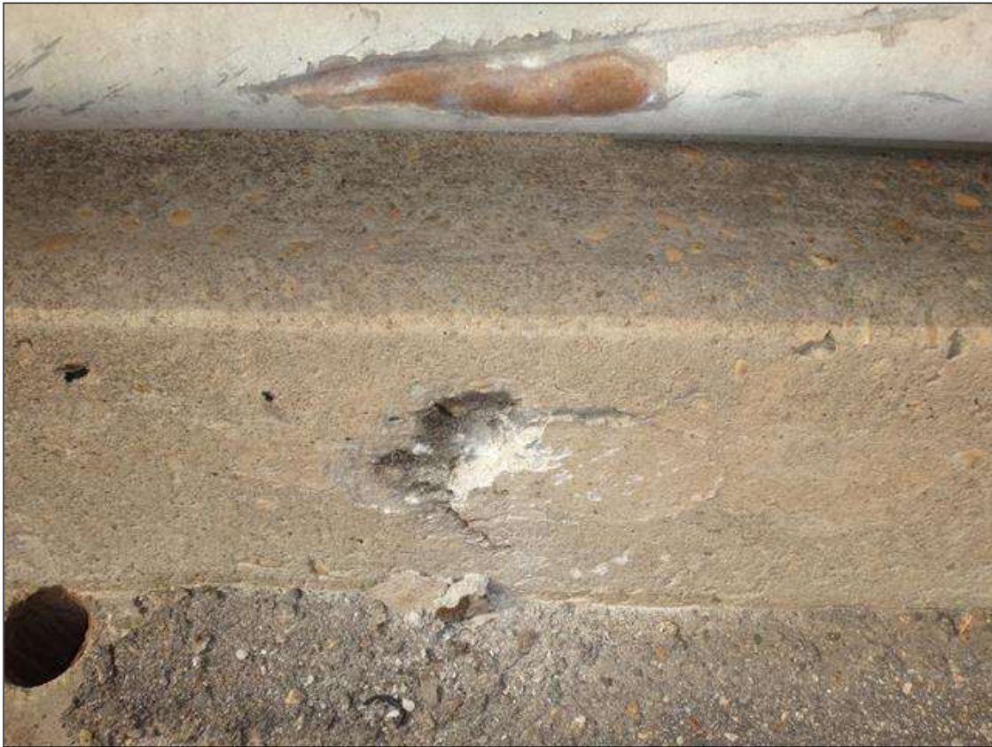
SPAN 3 SOUTH RAIL PARAPET, SPALL (3IN X 3IN X 1/4IN DEEP) WITH DELAMINATION (6IN X 3IN)
