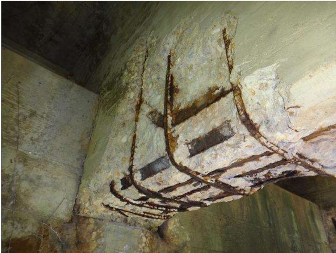
(PM) SPAN 2 BEAM 3 AT BENT 1, SPALL (33INX28INX2IN) WITH EXPOSED RUSTED REBAR, SECTION LOSS ON PRIMARY (NO MEASURABLE LOSS) AND SECONDARY (UP TO 50%)
