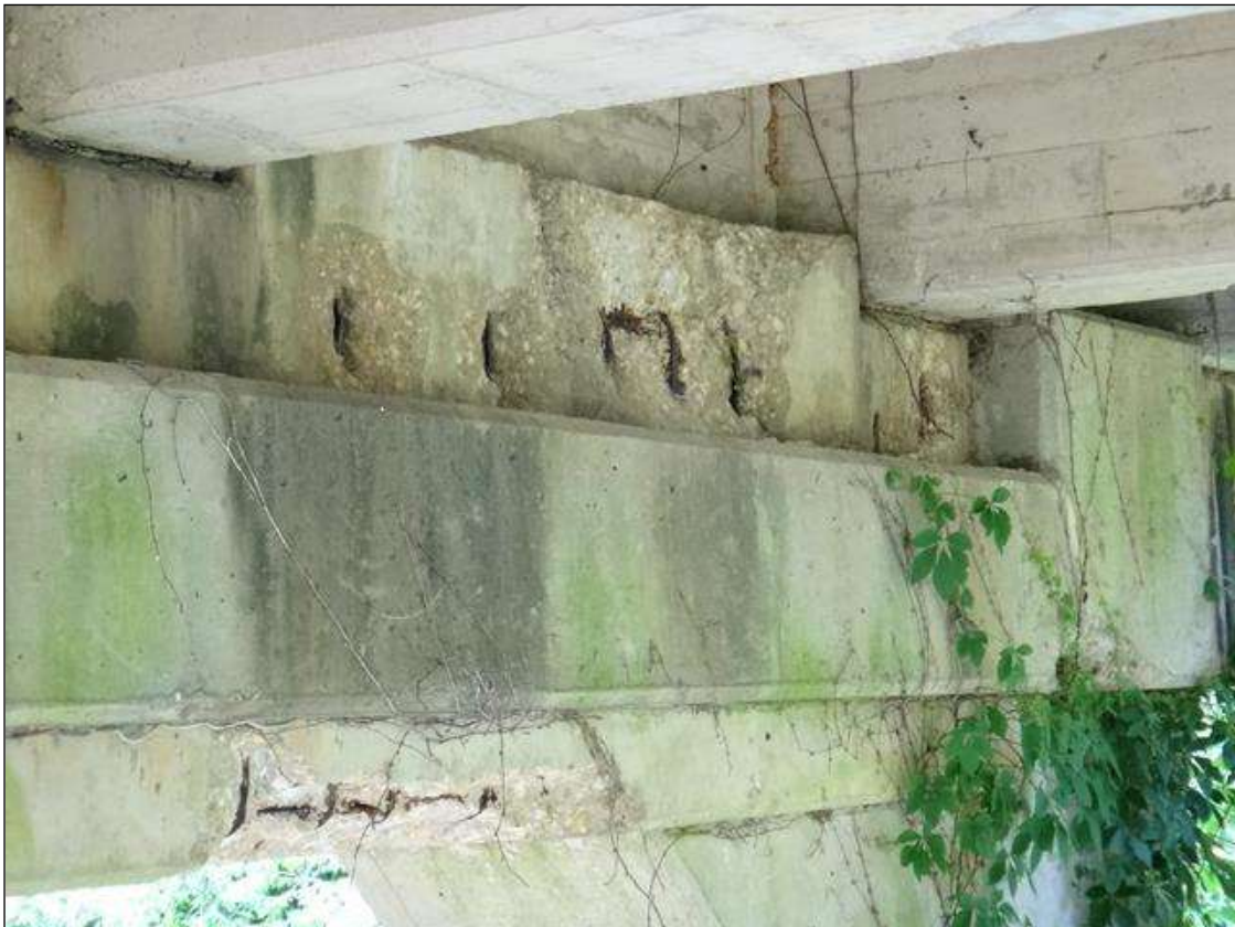
(PM) BENT 4 CAP WEST FACE, THREE (3) SPALLS (UP TO 4-1/2FT X 20IN X 3IN DEEP) WITH EXPOSED RUSTED REBAR, SECTION LOSS (NO MEASURABLE LOSS)
