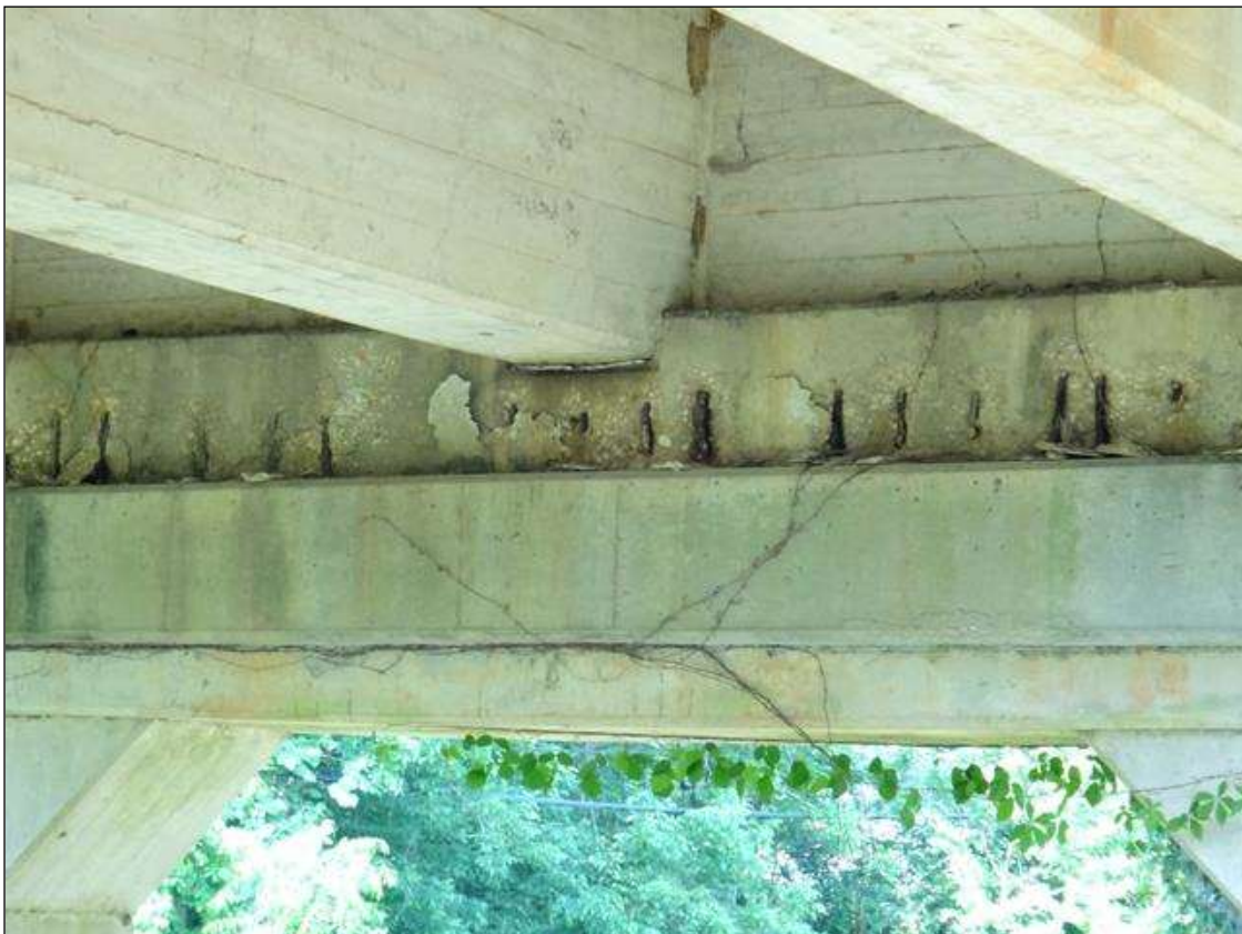
(PM) BEAM 5 CAP EAST FACE, MULTIPLE SPALLS (UP TO 20IN X 12IN)
