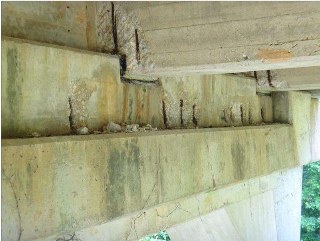
(PM) BENT 3 CAP WEST FACE, MULTIPLE SPALLS (UP TO 3FT X 10IN X 2IN DEEP) WITH EXPOSED RUSTED REBAR
