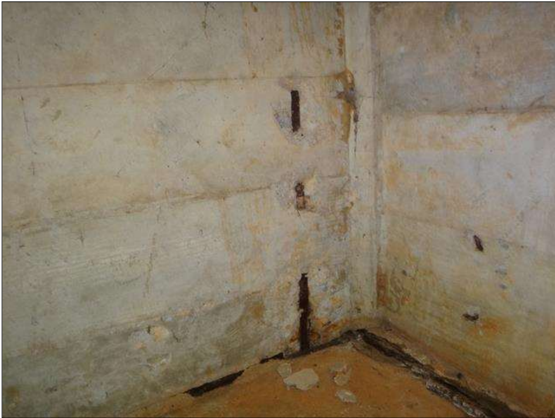
(PM) SPAN 10 BEAM 2 SOUTH FACE AT END BENT 2, THREE (3) SPALLS (UP TO 5IN X 3IN X 1IN DEEP) WITH EXPOSED RUSTED REBAR
