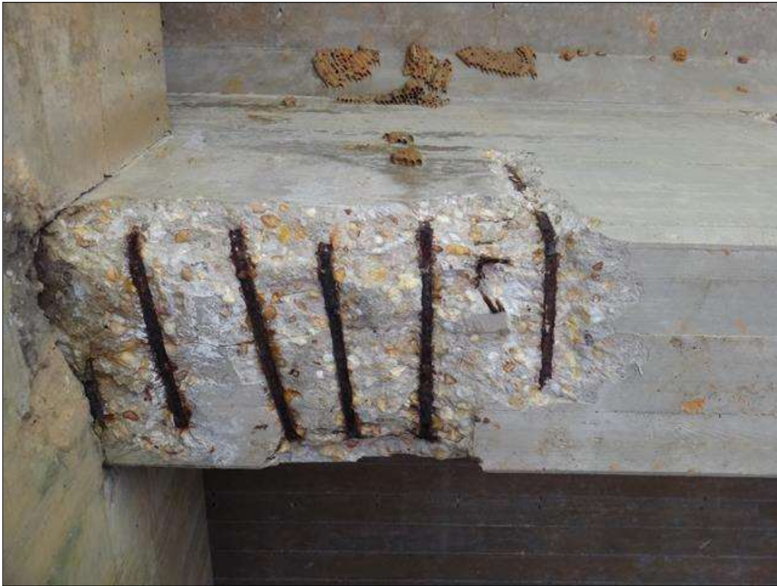
(PM) SPAN 1 BEAM 3 AT BENT 1, SPALL (30IN X 18IN X 2IN DEEP) WITH EXPOSED RUSTED REBAR, SECTION LOSS ON SECONDARY (UP TO 50%)
