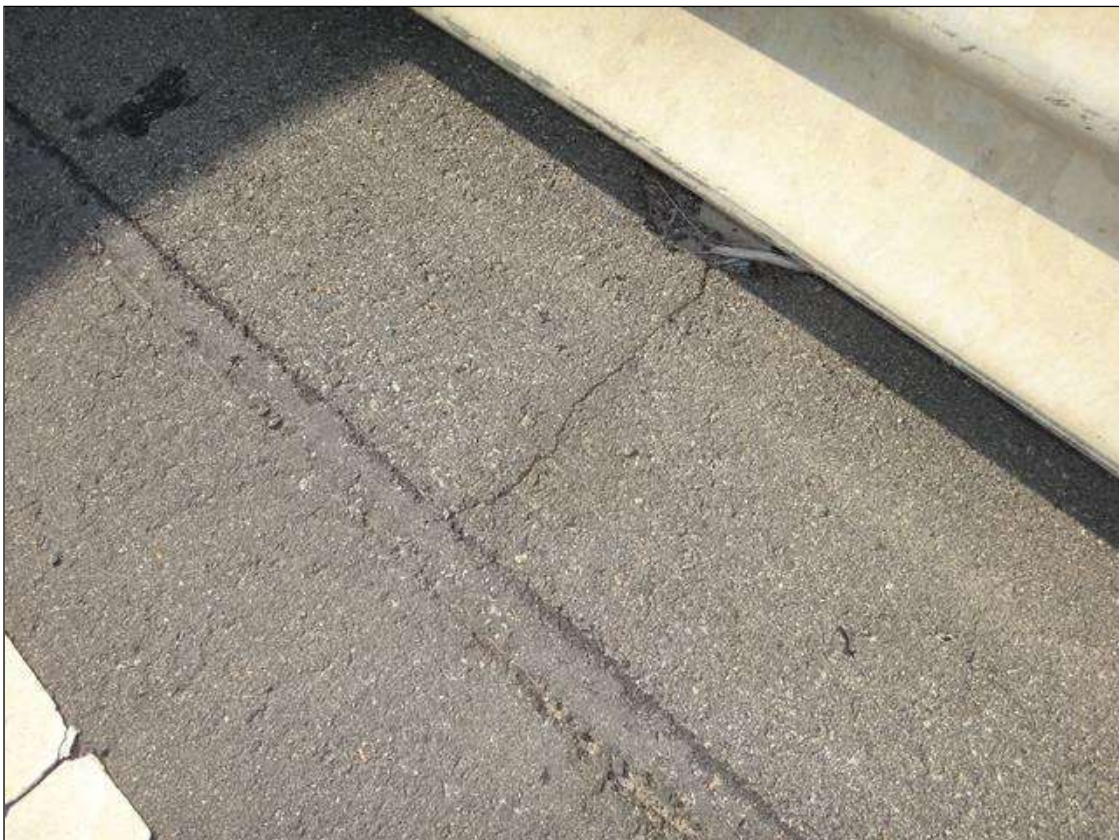
WEST APPROACH SOUTH SHOULDER ASPHALT WEARING SURFACE AT 15FT FROM END BENT 1, TRANSVERSE CRACK (1-1/2FT X 1/8IN)
