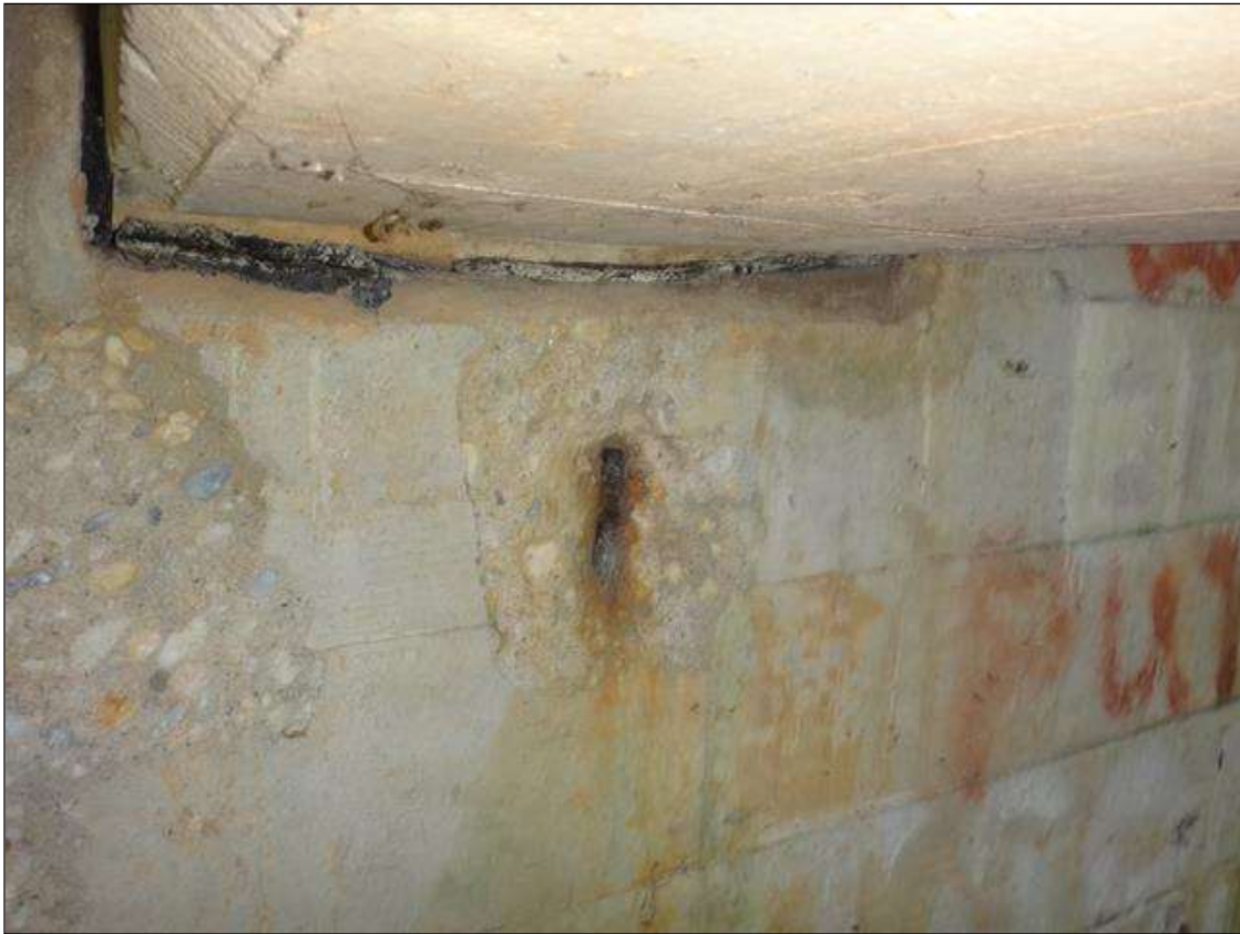
(PM) END BENT 2 CAP WEST FACE BELOW BEAM 3, SPALL (7IN DIAMETER X 1IN DEEP) WITH EXPOSED RUSTED REBAR
