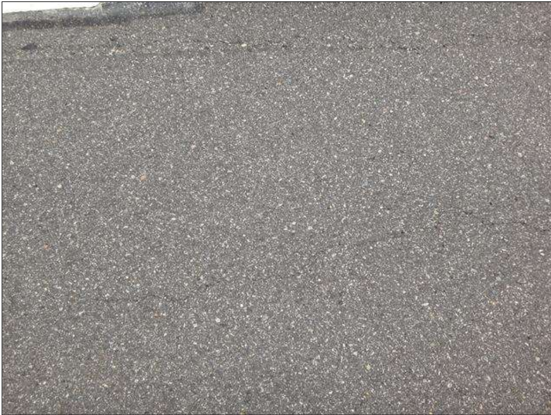
SPAN 1 ASPHALT WEARING SURFACE RIGHT LANE AT END BENT 1, LONGITUDINAL CRACK (6FT X 1/16IN)
