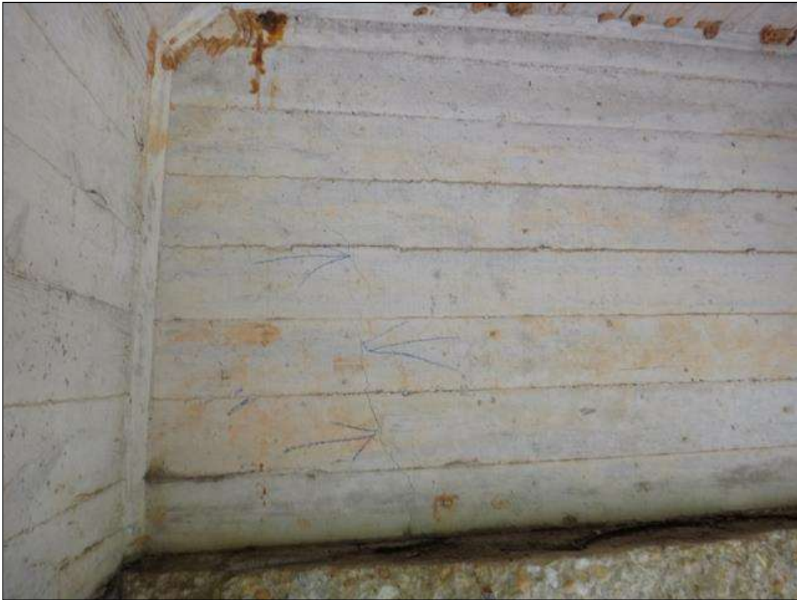
SPAN 5 BENT 4 BACKWALL AT BAY 2, VERTICAL CRACK (FULL HEIGHT X HAIRLINE)
