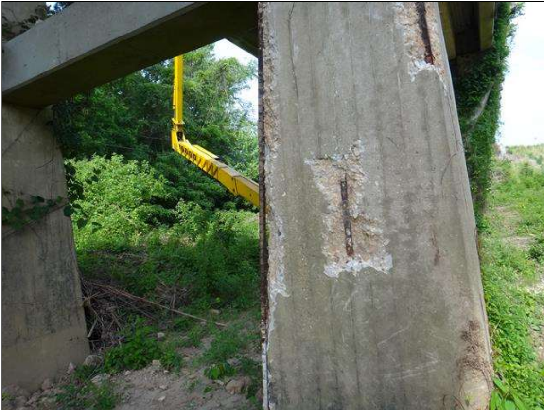
(PM) BENT 4 COLUMN 1 EAST FACE, THREE (3) SPALLS (UP TO 12FT X 14INX 4IN) WITH EXPOSED RUSTED REBAR, SECTION LOSS (NO MEASURABLE LOSS), DEBONDED REBAR
