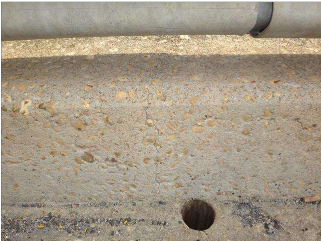
SPAN 1 NORTH RAIL PARAPET NEAR MIDSPAN, VERTICAL CRACK (3FT X 1/16IN) EXTENDS TO TOP SIDE
