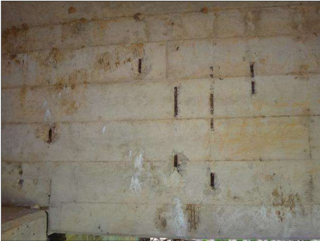
(PM) SPAN 10 BEAM 4 NORTH FACE AT 3FT FROM END BENT 2, SEVEN (7) SPALLS (UP TO 8IN X 3IN X 1/2IN DEEP) WITH EXPOSED RUSTED REBAR
