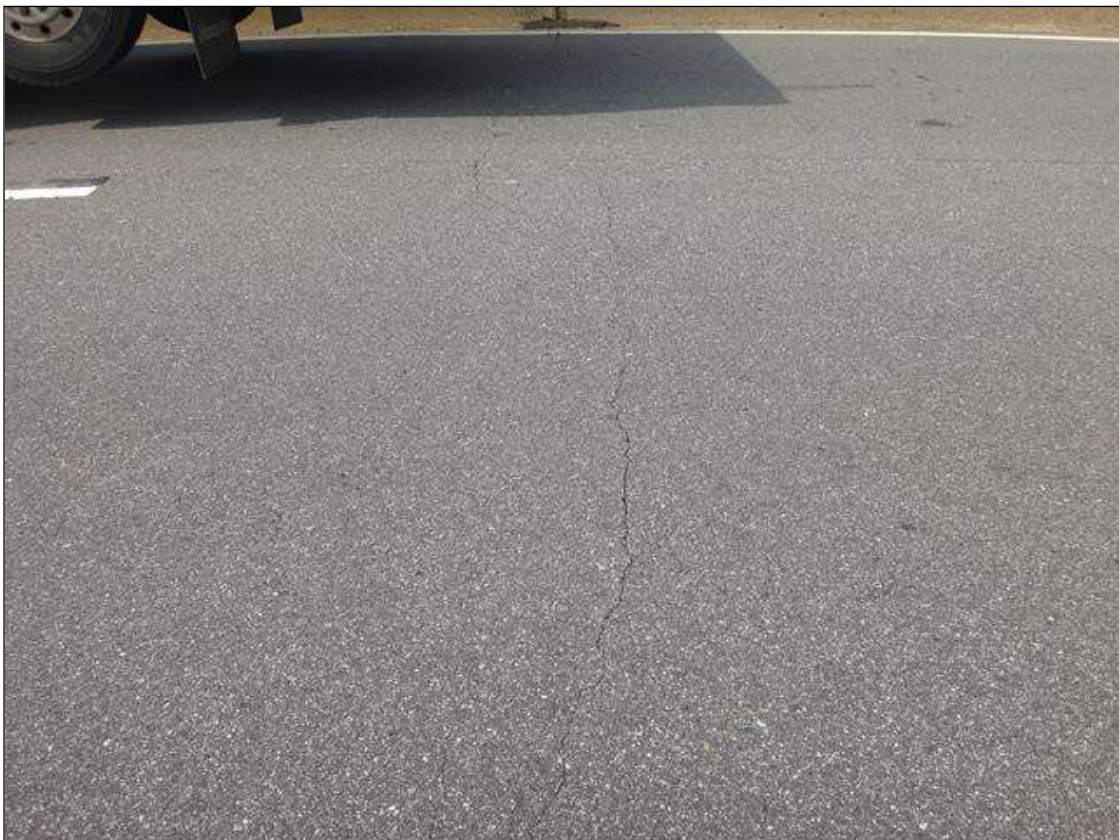
ASPHALT WEARING SURFACE OVER BENT 2, TWO (2) TRANSVERSE CRACKS (12FT X UP TO 1/4IN)
