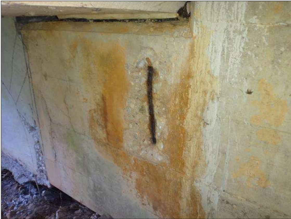
(PM) END BENT 2 CAP WEST FACE BELOW BEAM 2, SPALL (1FT X 6IN X 1IN DEEP) WITH EXPOSED RUSTED REBAR
