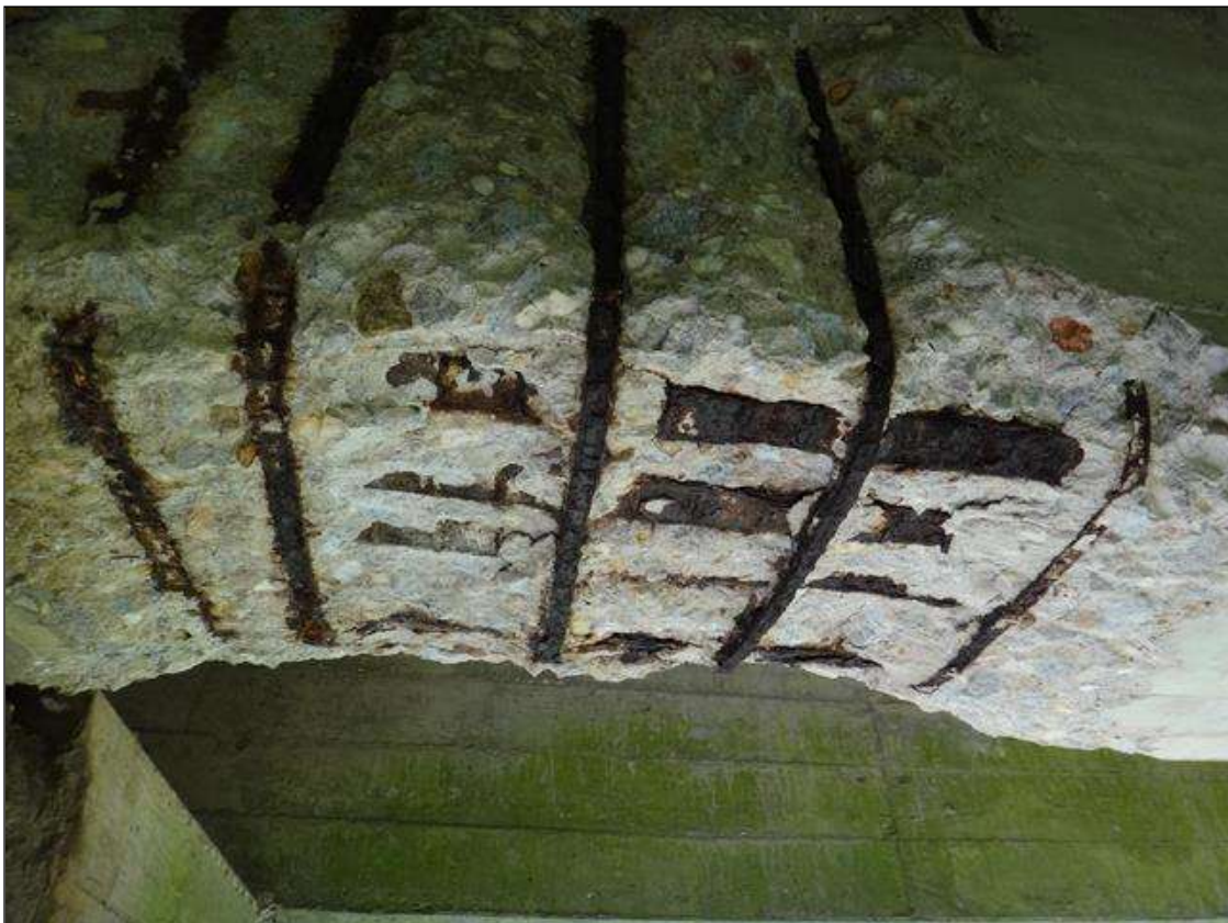
(PM) SPAN 2 BEAM 2 AT BENT 1, SPALL (48IN X 18IN X 2IN DEEP) WITH EXPOSED RUSTED REBAR
