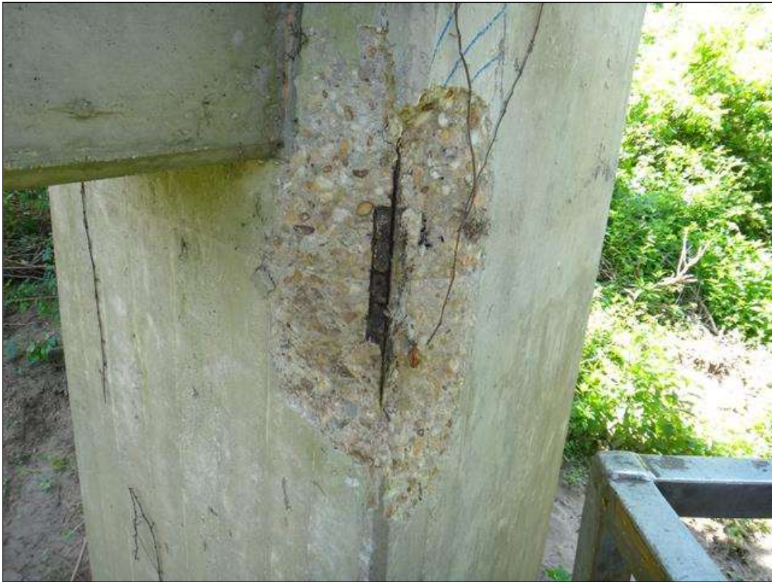
(PM) BENT 6 COLUMN 2 NORTHWEST CORNER, SPALL (2FT X 18IN X 3-1/2IN DEEP) WITH EXPOSED RUSTED REBAR, SECTION LOSS (NO MEASURABLE LOSS)
