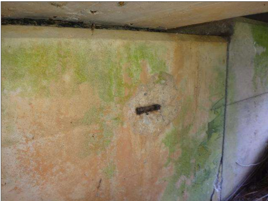
(PM) END BENT 1 CAP EAST FACE BELOW BEAM 2, SPALL (6IN X 4IN X 1/2IN DEEP) WITH EXPOSED RUSTED REBAR
