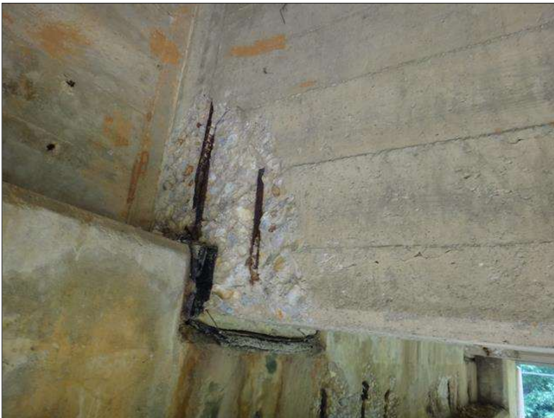
(PM) SPAN 3 BEAM 3 AT BENT 3, SPALL (16IN X 20IN X 2IN DEEP) WITH EXPOSED RUSTED REBAR, SECTION LOSS ON SECONDARY (50%)
