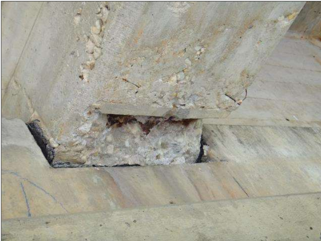
(PM) SPAN 2 BEAM 3 AT BENT 2, SPALL (18IN X 8IN X 3IN DEEP) WITH EXPOSED RUSTED REBAR
