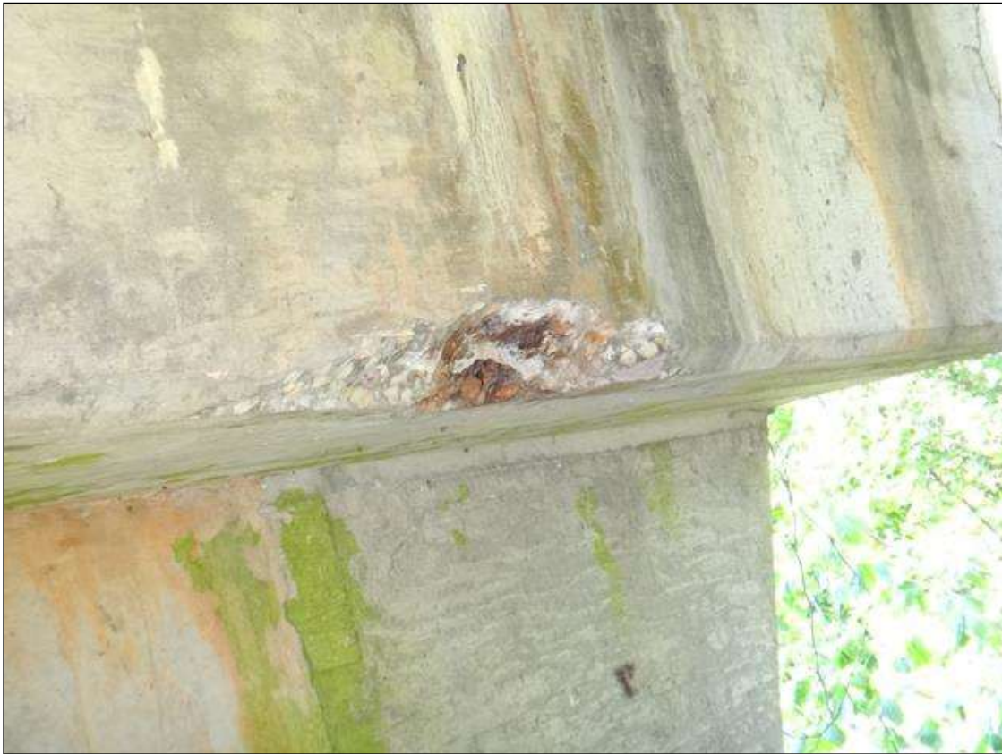
(PM) BENT 1 CAP WEST FACE BELOW BENT 4, SPALL (20IN X 6IN X 3IN DEEP) WITH EXPOSED RUSTED REBAR
