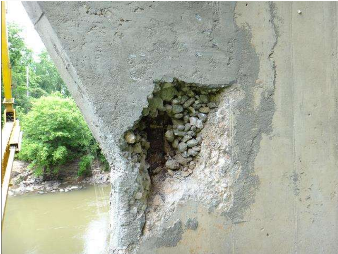
(PM) BENT 9 COLUMN 2 SOUTHEAST CORNER, SPALL (11IN X 8IN X 3IN DEEP) WITH EXPOSED RUSTED REBAR
