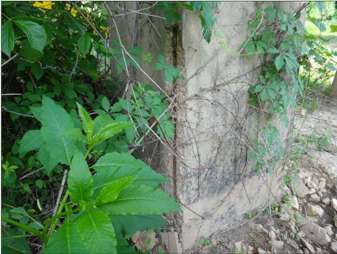
(PM) BENT 4 COLUMN 2 SOUTHEAST CORNER, SPALL (6FT X 8IN X 2IN DEEP) WITH EXPOSED RUSTED REBAR, SECTION LOSS (NO MEASURABLE LOSS)
