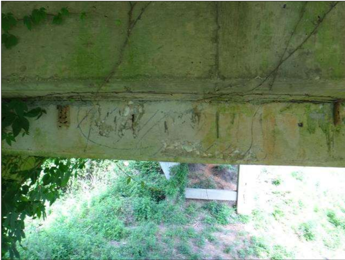
BENT 2 CAP EAST FACE BELOW BEAM 3, DELAMINATION/SPALL (30IN X 8IN X 1IN DEEP) WITH EXPOSED RUSTED REBAR
