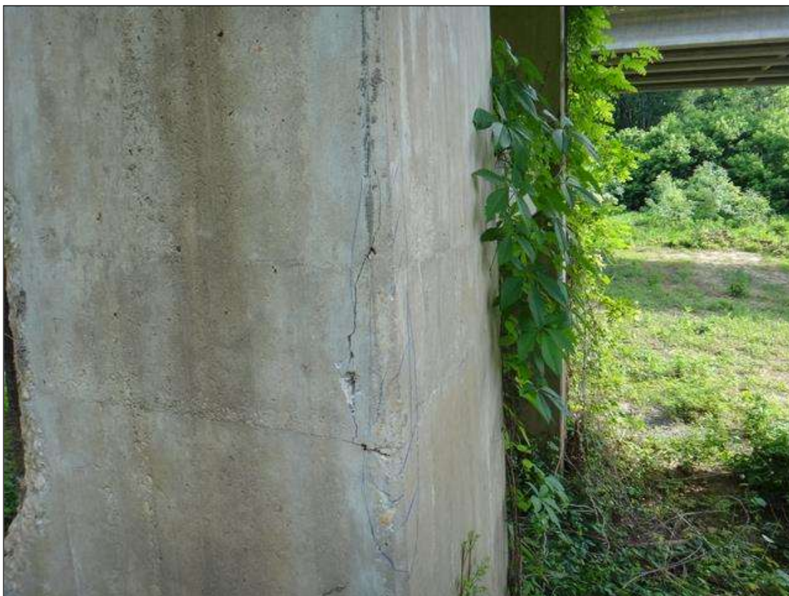
BENT 3 COLUMN 2 SOUTHEAST CORNER, DELAMINATION (2FT X 4IN)
