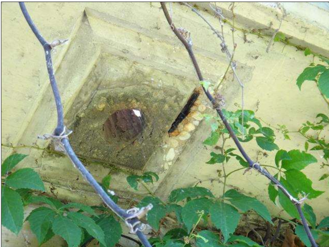
SPAN 7 NORTH OVERHANG AT SCUPPER 1, SPALL (12IN X 4IN X 1IN DEEP) WITH EXPOSED RUSTED REBAR
