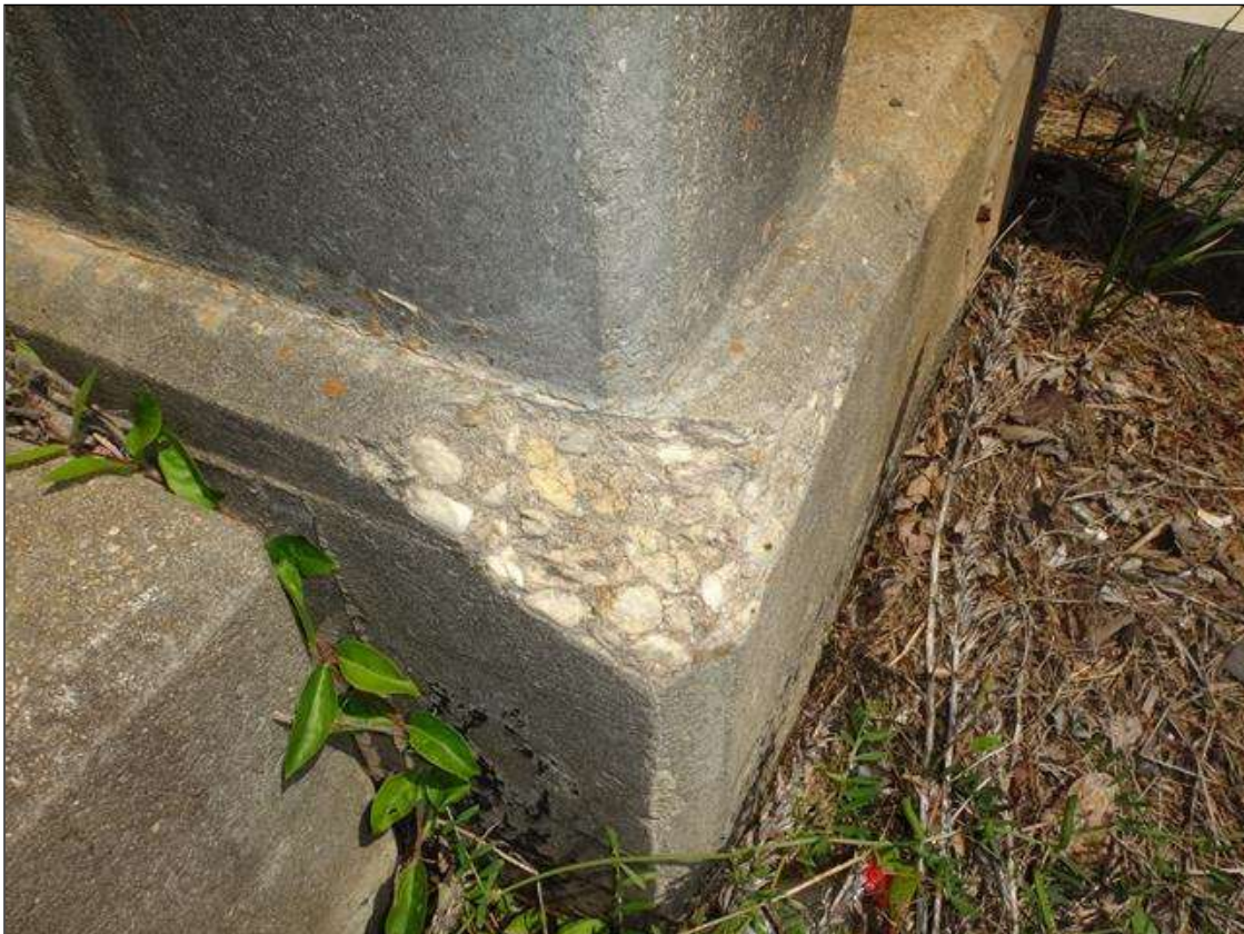
SOUTH RAIL END POST BASE AT END BENT 2, SPALL (6IN X 4IN X 1IN DEEP)
