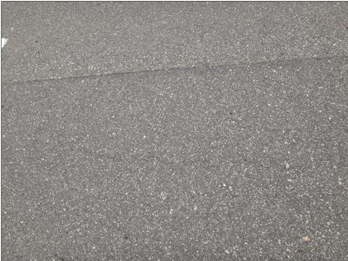
SPAN 10 ASPHALT WEARING SURFACE RIGHT LANE AT END BENT 2, LONGITUDINAL CRACK (8FT X 1/16IN)
