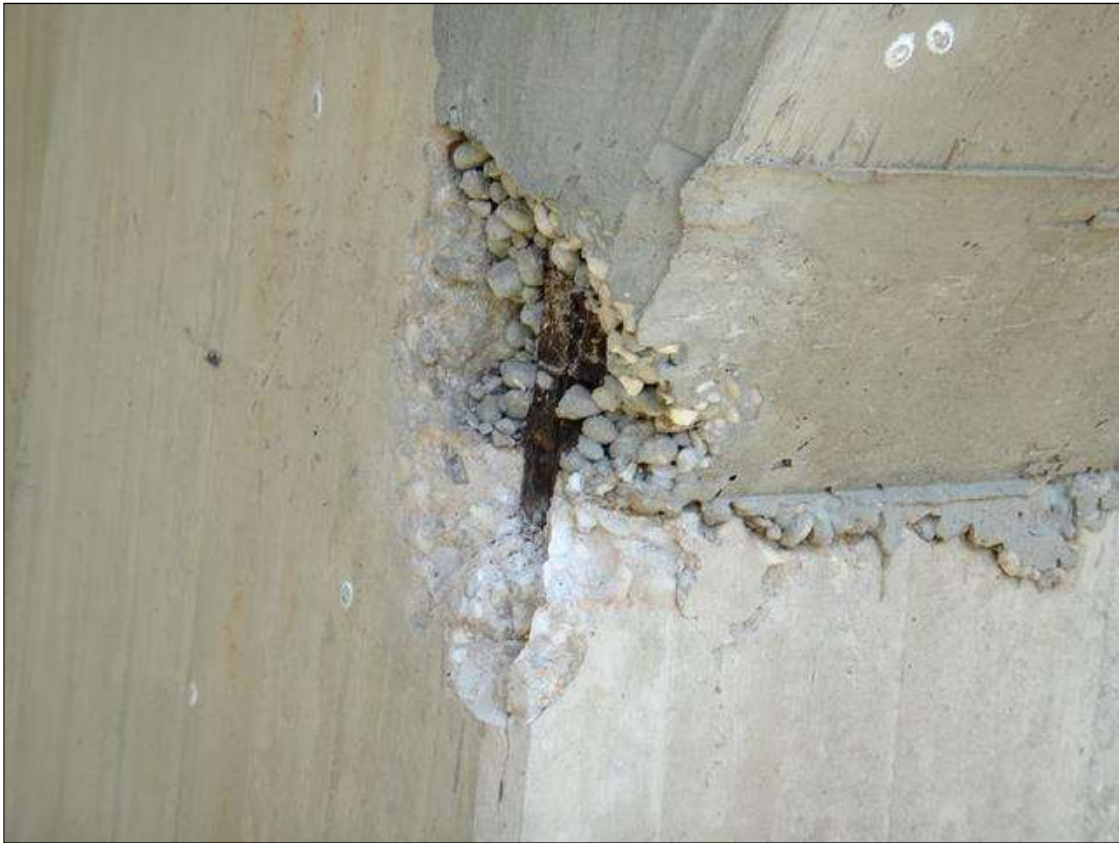
(PM) BENT 8 COLUMN 2 SOUTHWEST CORNER, SPALL (16IN X 8IN X 3IN DEEP) WITH EXPOSED RUSTED REBAR, SECTION LOSS (NO MEASURABLE LOSS)
