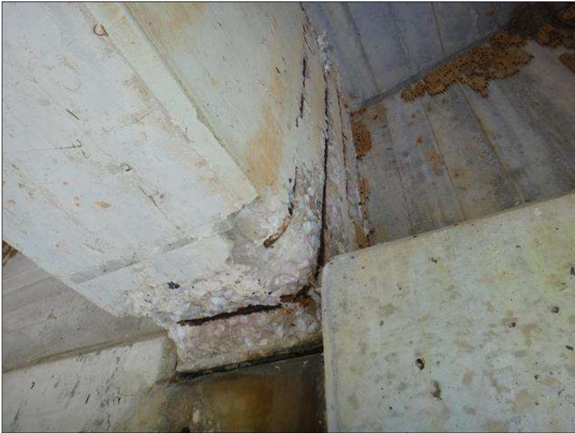
(PM) SPAN 9 BEAM 4 AT BENT 9, SPALL (18IN X 48IN X 3-1/2IN DEEP) WITH EXPOSED RUSTED REBAR, SECTION LOSS (NO MEASURABLE LOSS)
