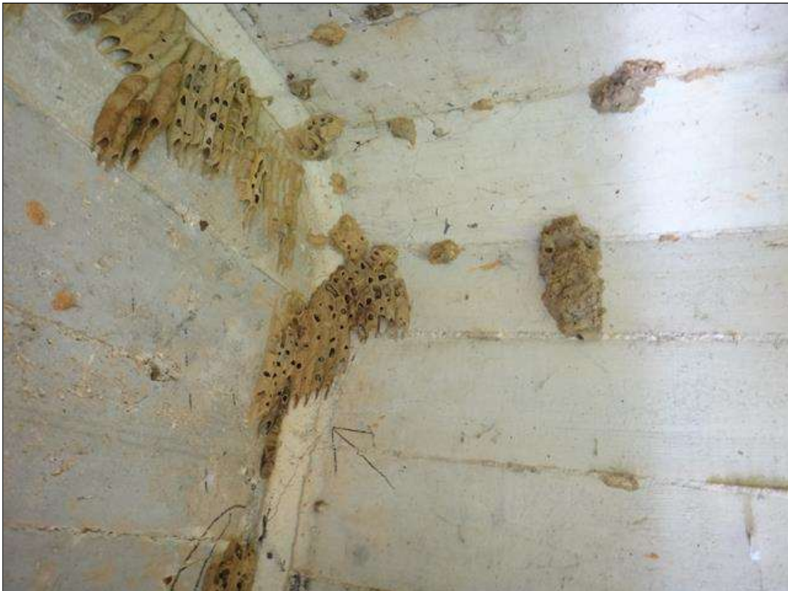
SPAN 9 BEAM 3 AT BENT 8, DIAGONAL CRACK (24IN X 1/64IN) EXTENDS INTO DECK (2FT)
