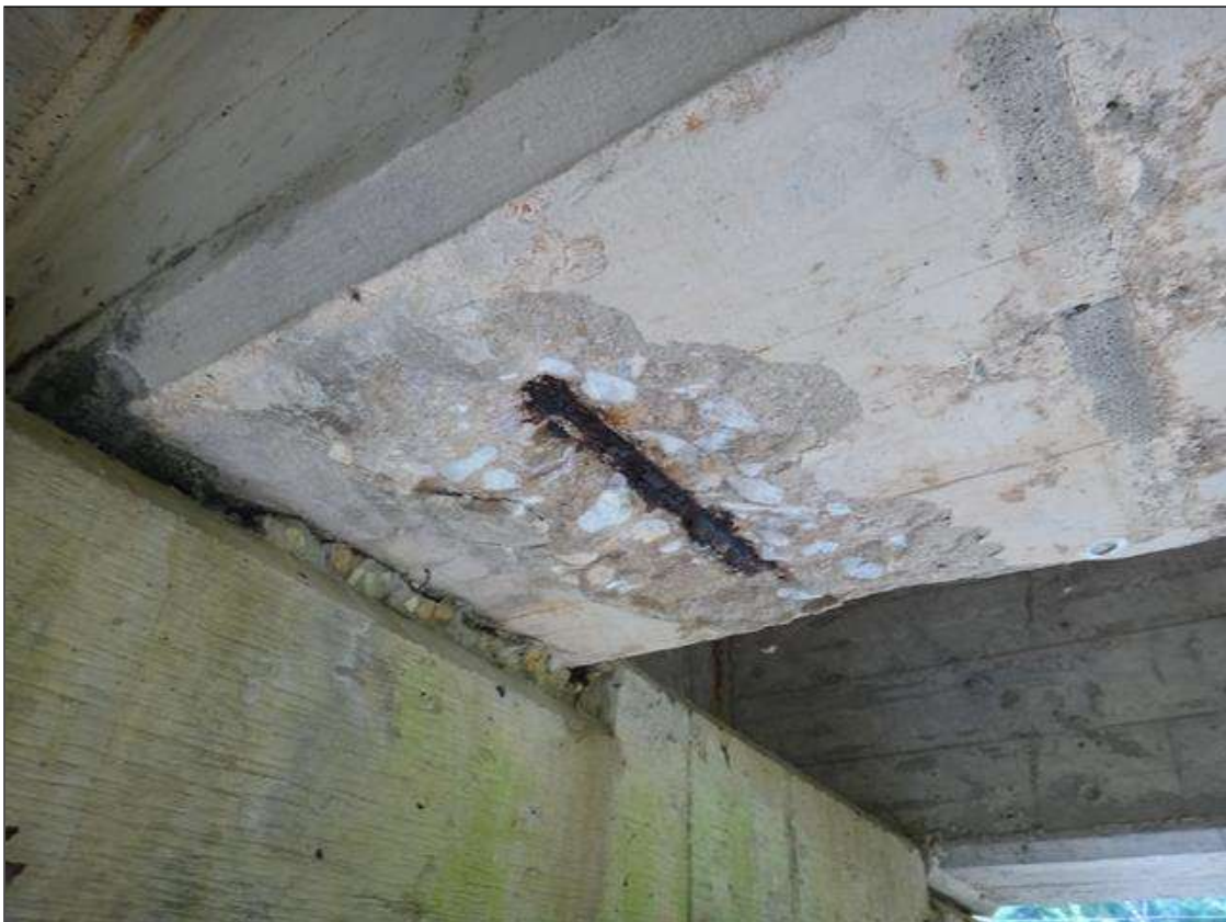
(PM) SPAN 8 BEAM 4 AT BENT 8, SPALL (16IN X 8IN X 1-1/2IN DEEP) WITH EXPOSED RUSTED REBAR
