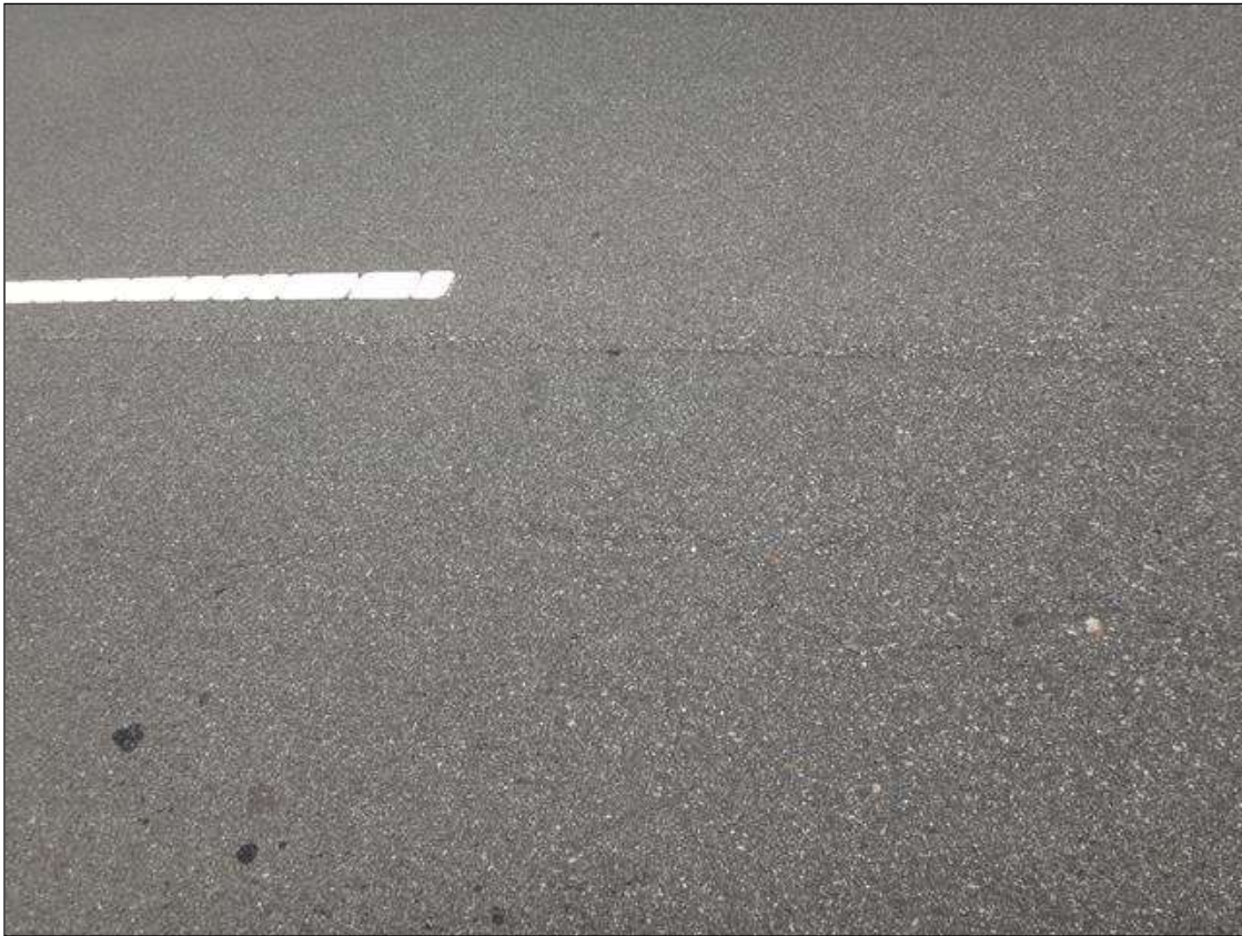
SPAN 7 ASPHALT WEARING SURFACE RIGHT LANE AT 3FT FROM BENT 7, LONGITUDINAL CRACK (10FT X 1/16IN)
