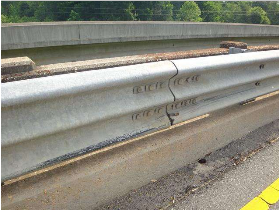
SPAN 1 NORTH RAIL AT 10FT FROM BENT 1, IMPACT SCRAPES (8FT)
