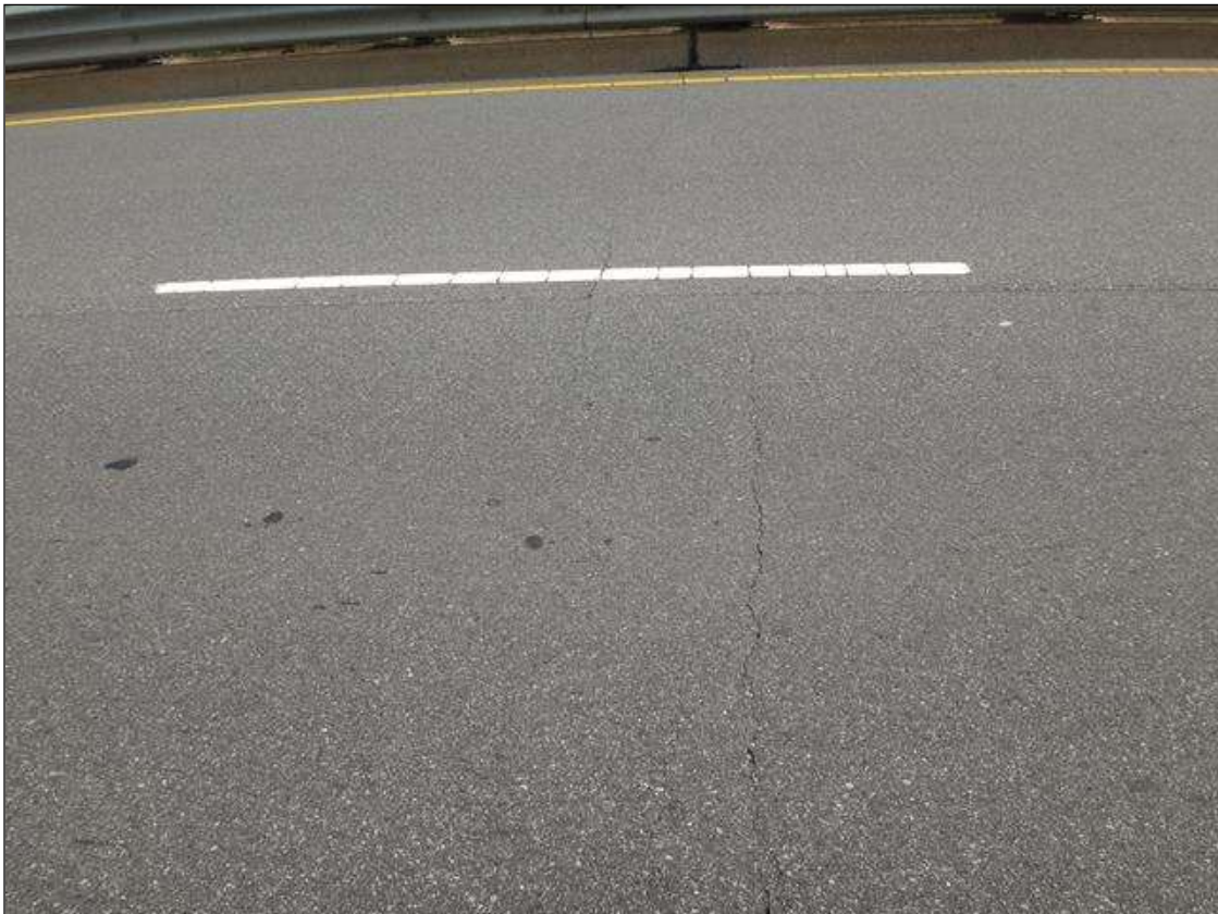
ASPHALT WEARING SURFACE OVER BENT 6, TWO (2) TRANSVERSE CRACKS (13FT X 1/8IN)
