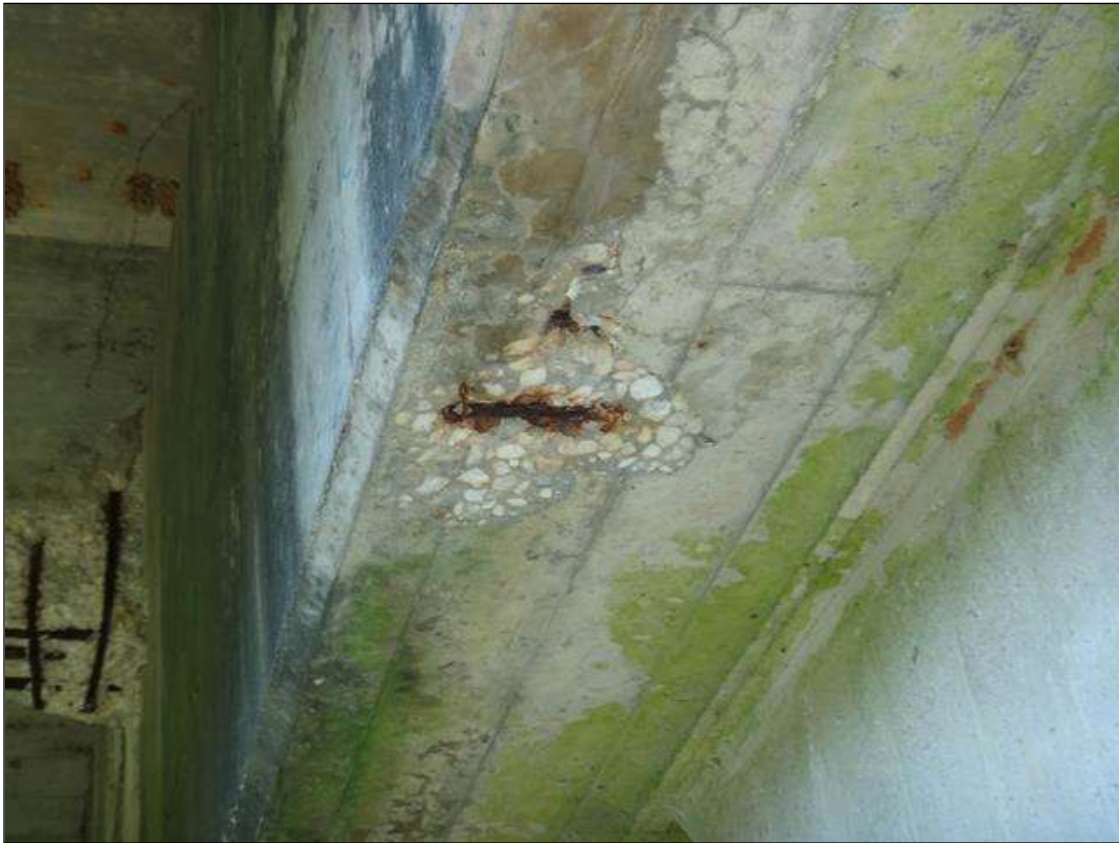
(PM) BENT 1 CAP UNDERSIDE BELOW BEAM 2, SPALL (12IN X 12IN X 1IN DEEP) WITH EXPOSED RUSTED REBAR
