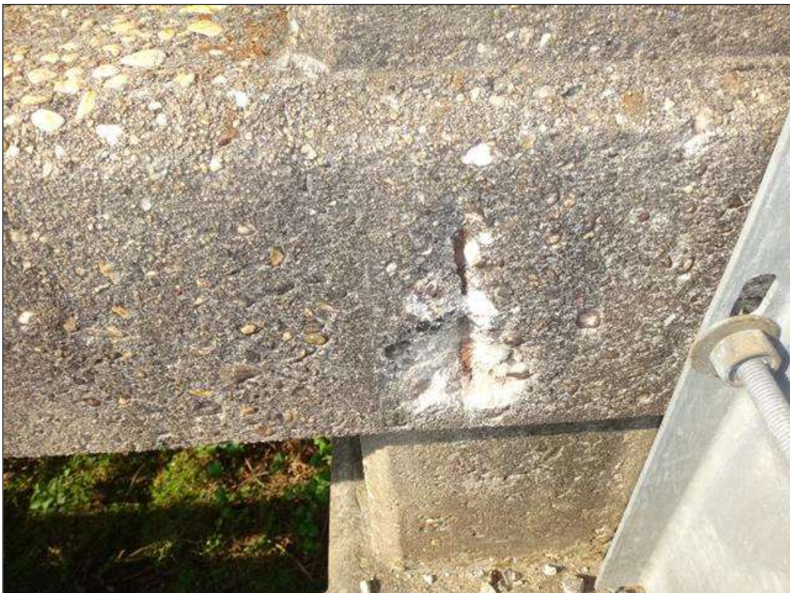
SPAN 1 SOUTH RAIL AT 20FT FROM END BENT 1, SPALL (6IN X 3IN X 1/2IN DEEP)
