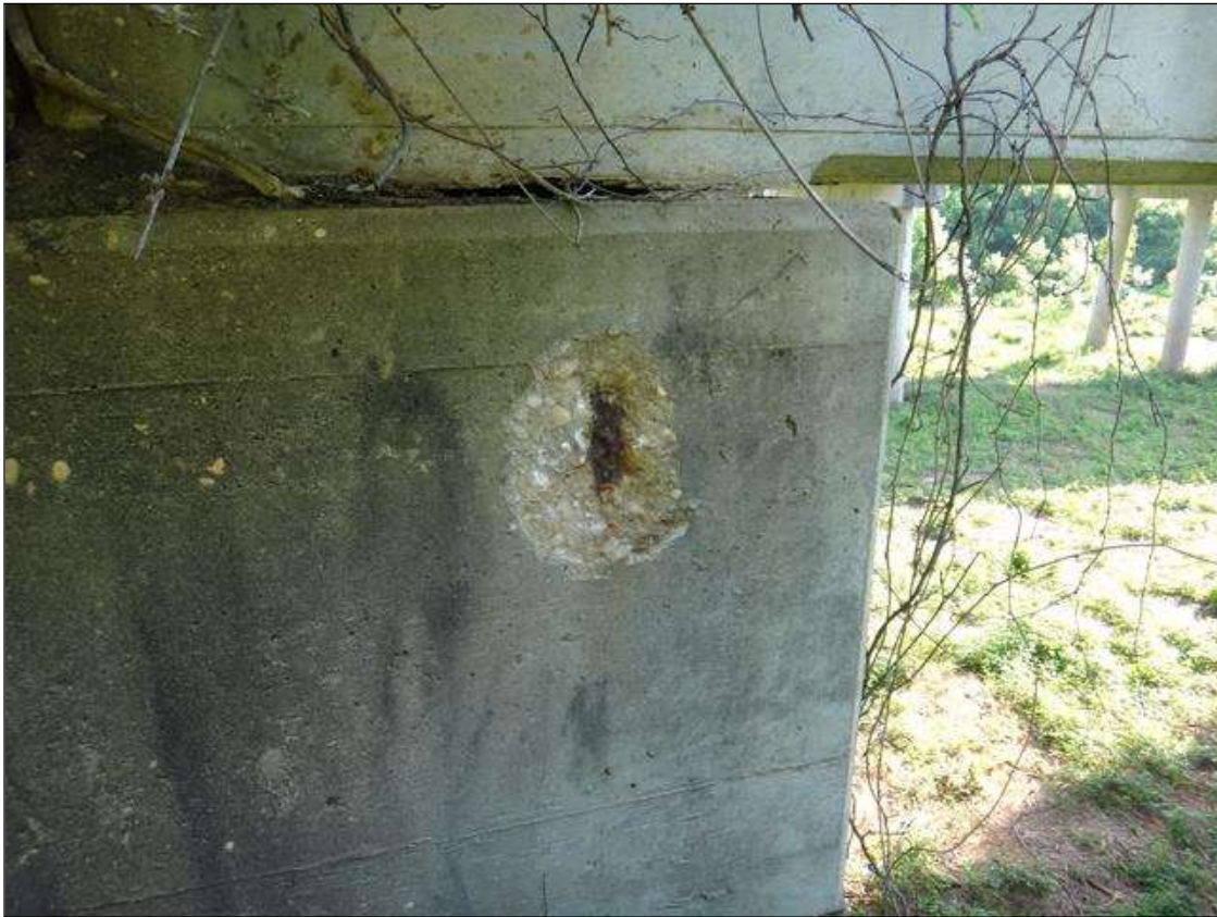
(PM) BENT 1 CAP SOUTH FACE, SPALL (12IN X 7IN X 1IN DEEP) WITH EXPOSED RUSTED REBAR
