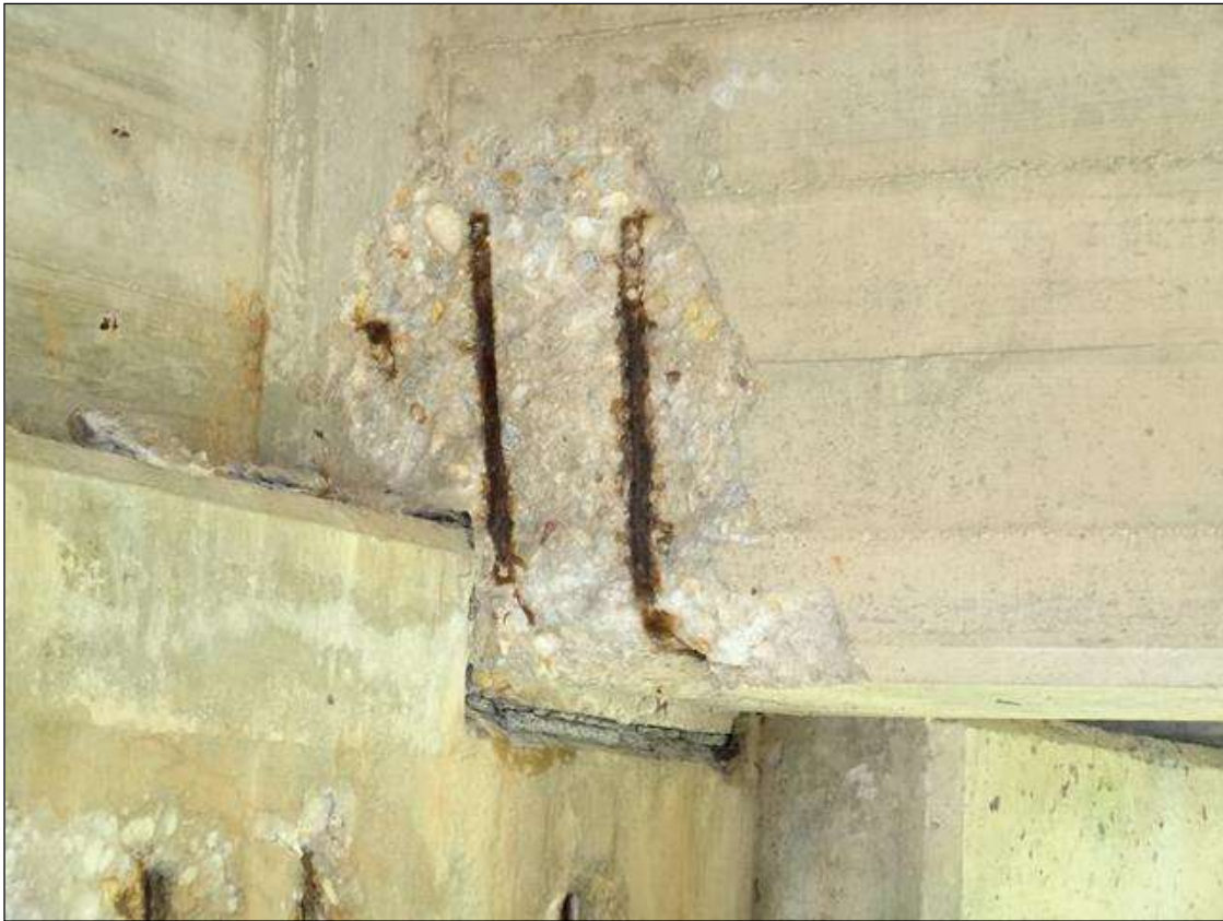
(PM) SPAN 3 BEAM 4 AT BENT 3, SPALL (20IN X 20IN X 2IN DEEP) WITH EXPOSED RUSTED REBAR, SECTION LOSS (NO MEASURABLE LOSS)
