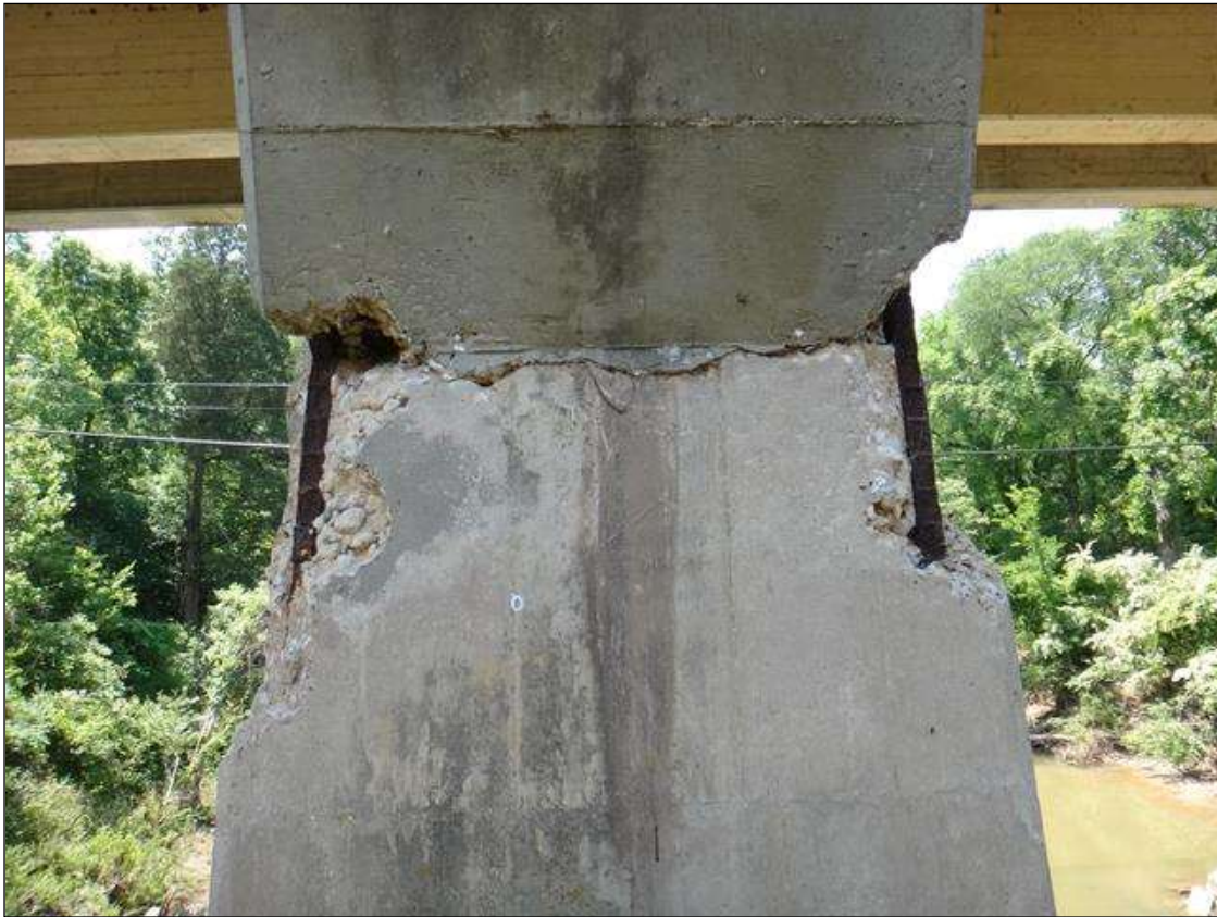
(PM) BENT 8 COLUMN 1 NORTH FACE, TWO (2) SPALLS (2FT X 8IN X 4IN DEEP) WITH EXPOSED RUSTED REBAR, SECTION LOSS (NO MEASURABLE LOSS) AND DEBONDED REBAR
