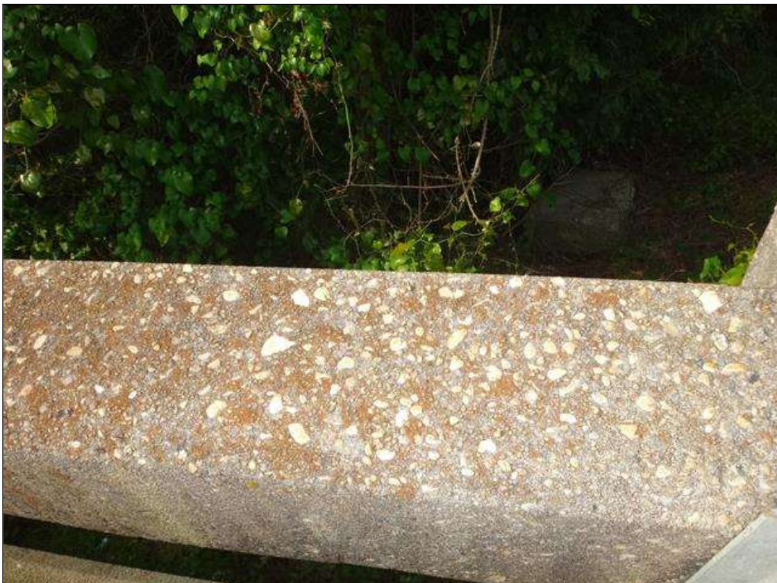
SOUTH RAIL, SCALING WITH EXPOSED AGGREGATE
