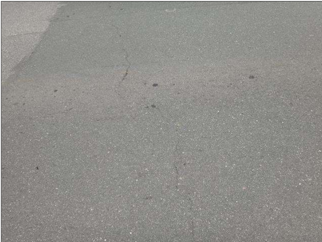
EAST APPROACH ASPHALT WEARING SURFACE AT 3FT FROM END BENT 2, TRANSVERSE CRACK (20FT X UP TO 1/4IN)
