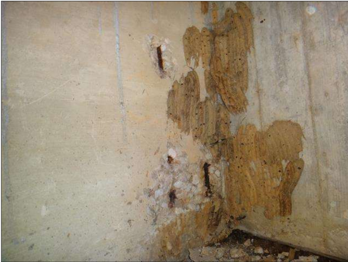
(PM) SPAN 8 BEAM 2 AT BENT 7, TWO (2) SPALLS (UP TO 12IN X 8IN X 1IN DEEP) WITH EXPOSED RUSTED REBAR
