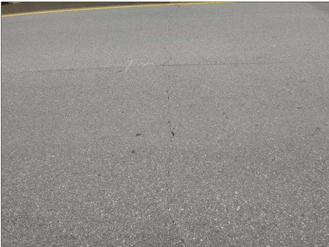
ASPHALT WEARING SURFACE OVER END BENT 2, TRANSVERSE CRACK (FULL WIDTH X UP TO 1/4IN)
