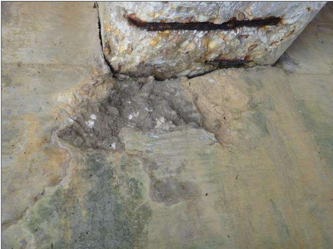
BENT 1 CAP WEST FACE BELOW BENT 3, SPALL (20IN X 9IN X 2-1/2IN DEEP)
