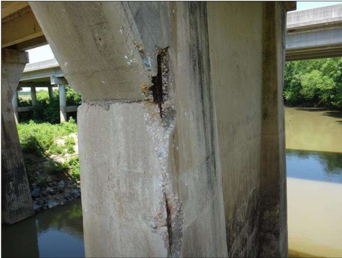
(PM) BENT 8 COLUMN 2 SOUTHEAST CORNER AT 10FT BELOW CAP, SPALL (6FT X 1FT X 5IN DEEP) WITH EXPOSED RUSTED REBAR, SECTION LOSS (NO MEASURABLE LOSS)
