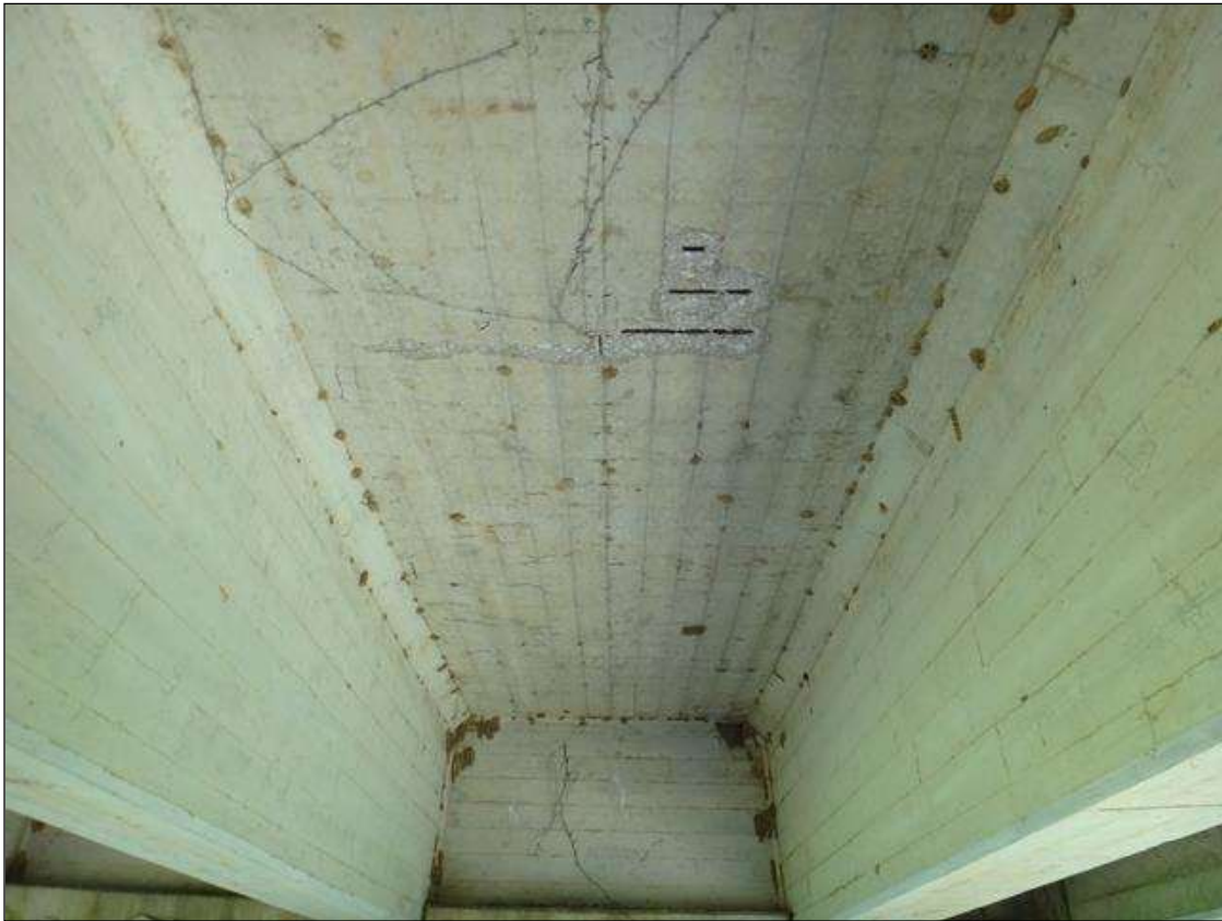
SPAN 7 UNDERSIDE OF DECK AT BAY 2, MULTIPLE SPALLS (UP TO 4FT X 2FT X 2IN DEEP) WITH EXPOSED RUSTED REBAR, SECTION LOSS (NO MEASURABLE LOSS)
