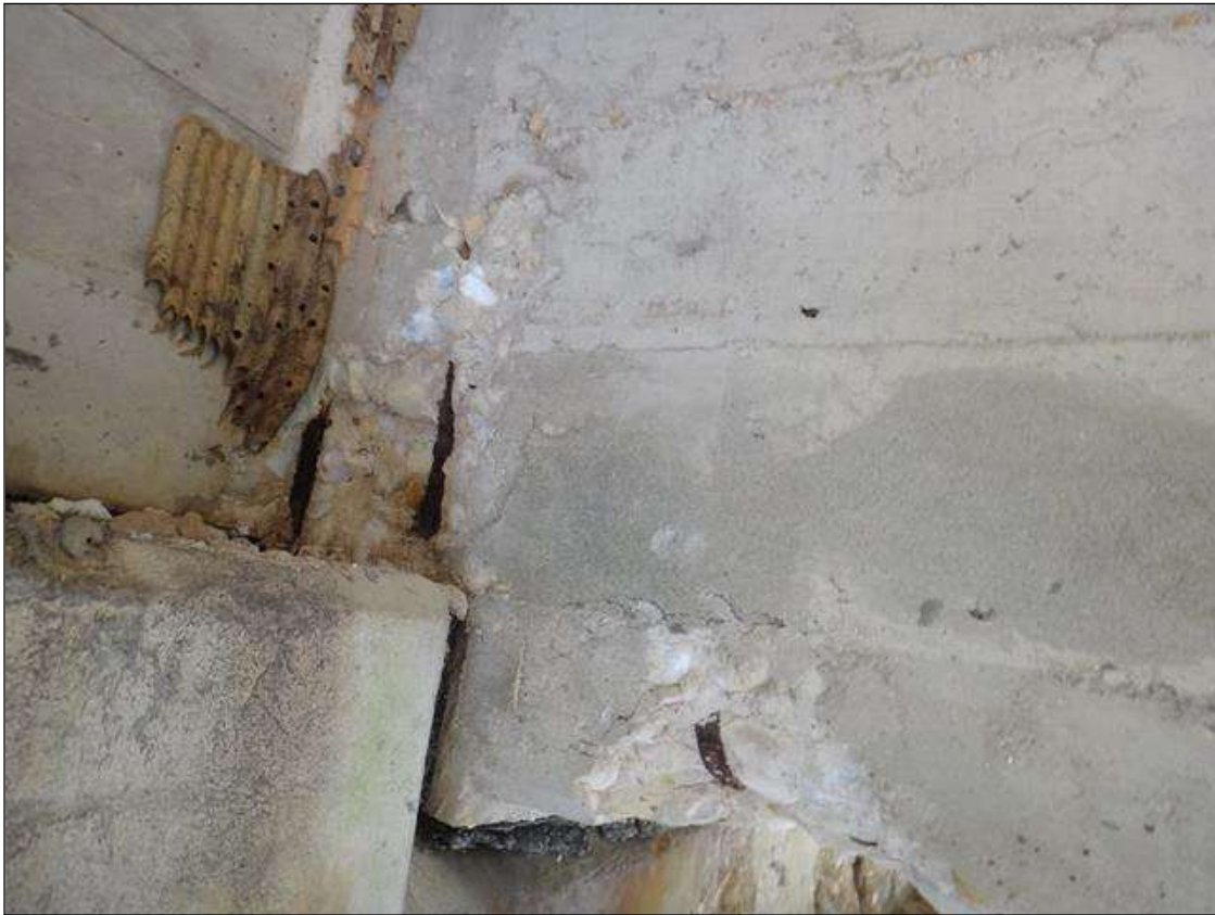
(PM) SPAN 9 BEAM 3 NORTH FACE AT BENT 9, TWO (2) SPALLS (UP TO 12IN X 6IN X 2IN DEEP) WITH EXPOSED RUSTED REBAR
