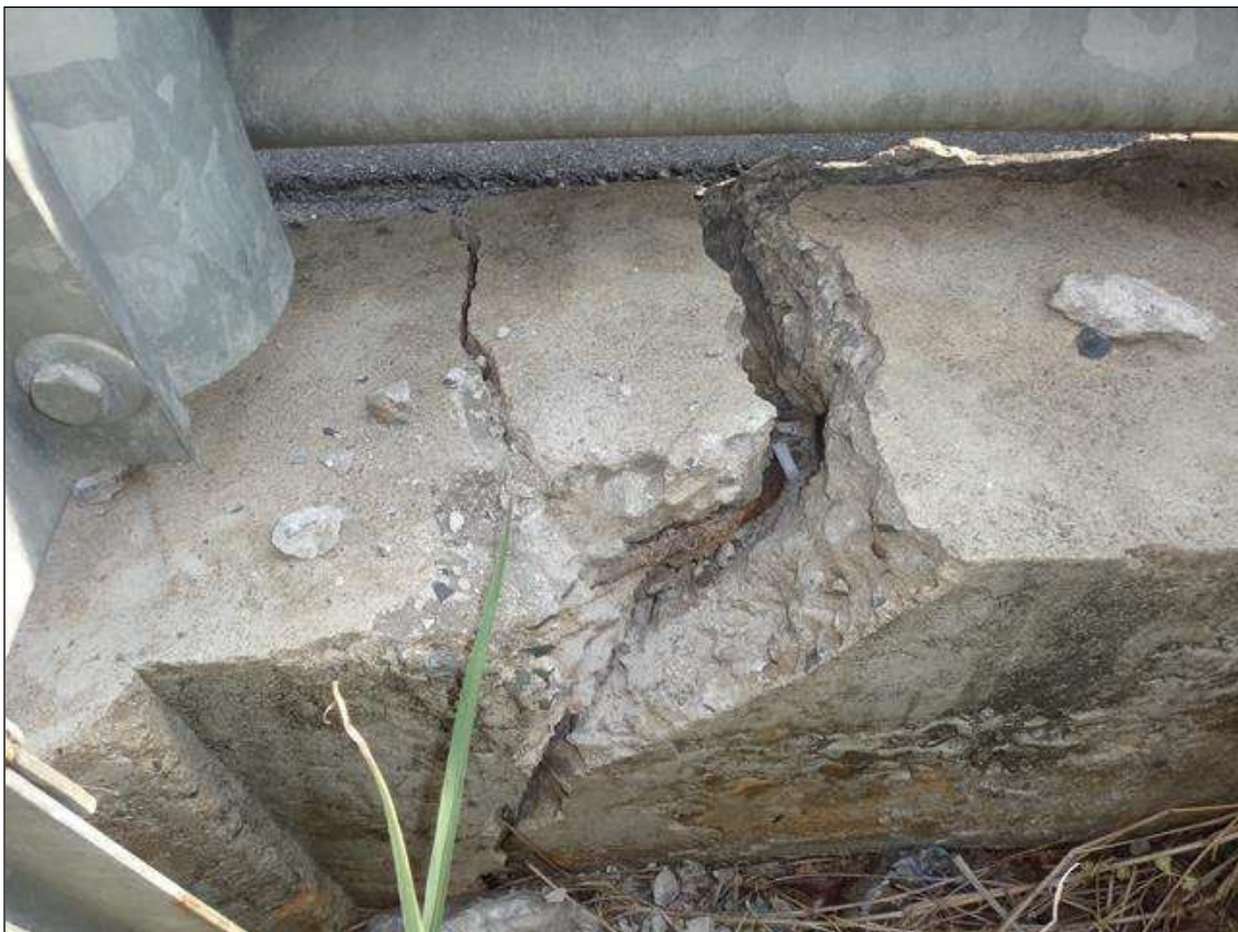
WEST APPROACH SOUTH CURB AT END BENT 1, BROKEN WITH SPALL (4IN X 8IN X 6IN DEEP) WITH EXPOSED RUSTED REBAR
