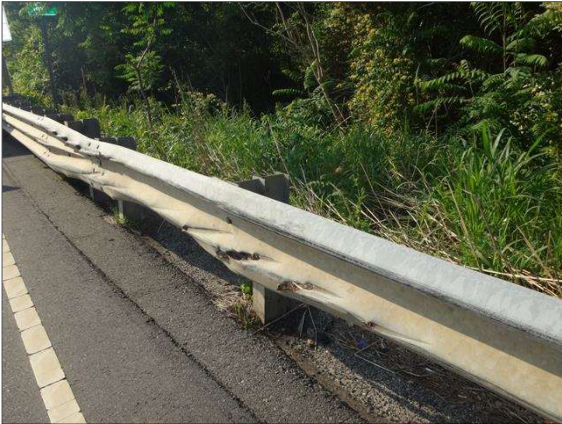
SOUTHWEST GUARDRAIL AT 20FT FROM END BENT 1, IMPACT DAMAGE (17FT)
