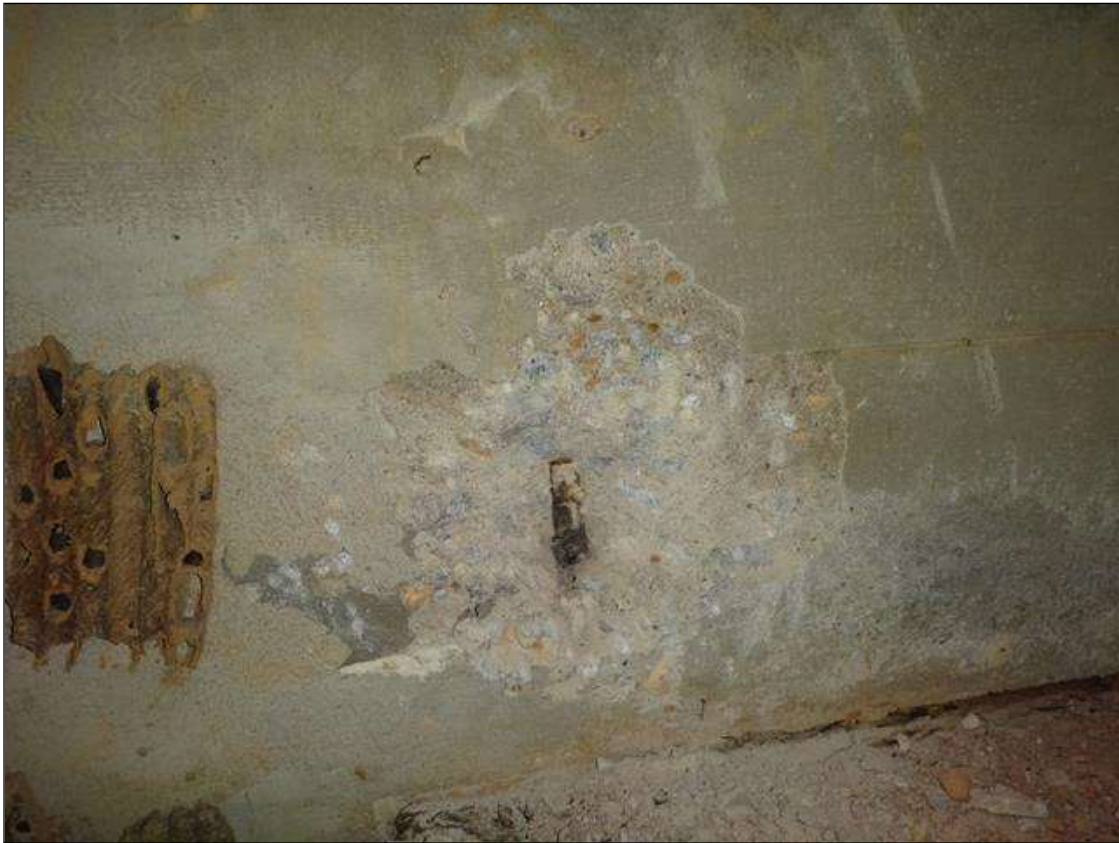
(PM) SPAN 1 BEAM 3 NORTH FACE AT END BENT 1, SPALL (10IN X 8IN X 2IN DEEP) WITH EXPOSED RUSTED REBAR
