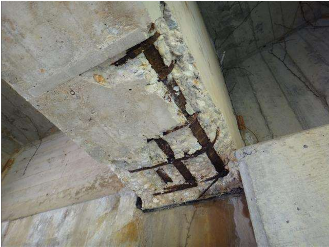
(PM) SPAN 2 BEAM 4 AT BENT 2, SPALL (30INX18INX4IN) WITH EXPOSED RUSTED REBAR, SECTION LOSS ON PRIMARY (NO MEASURABLE LOSS) AND SECONDARY (UP TO 100%)
