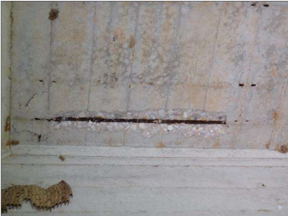
SPAN 5 BENT 5 UNDERSIDE OF DECK AT BAY 2, SPALL (3FT X 4IN X 1IN DEEP) WITH EXPOSED RUSTED REBAR AND ADJACENT DELAMINATION
