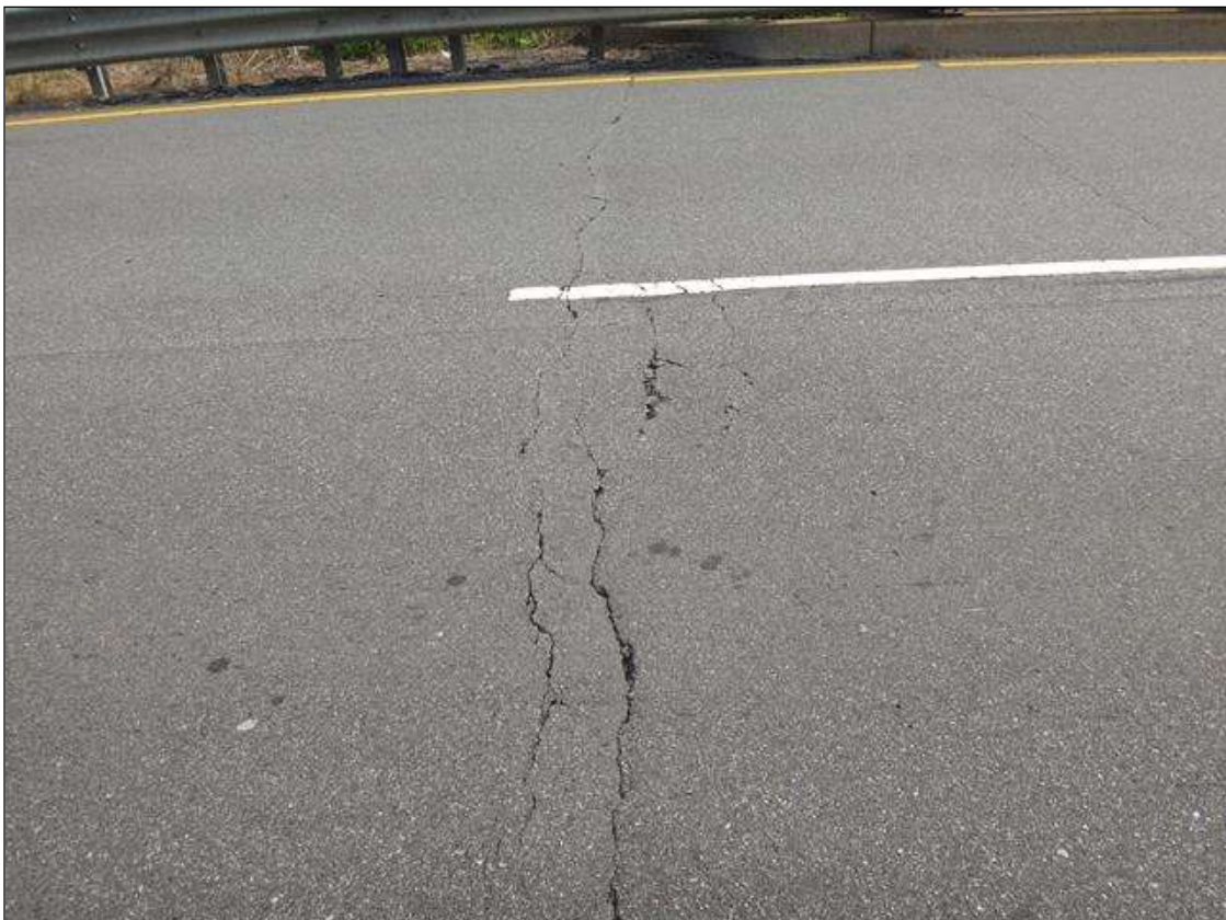
WEST APPROACH ASPHALT WEARING SURFACE AT 5FT FROM END BENT 1, FOUR (4) TRANSVERSE CRACKS (UP TO FULL WIDTH X UP TO 1/2IN)
