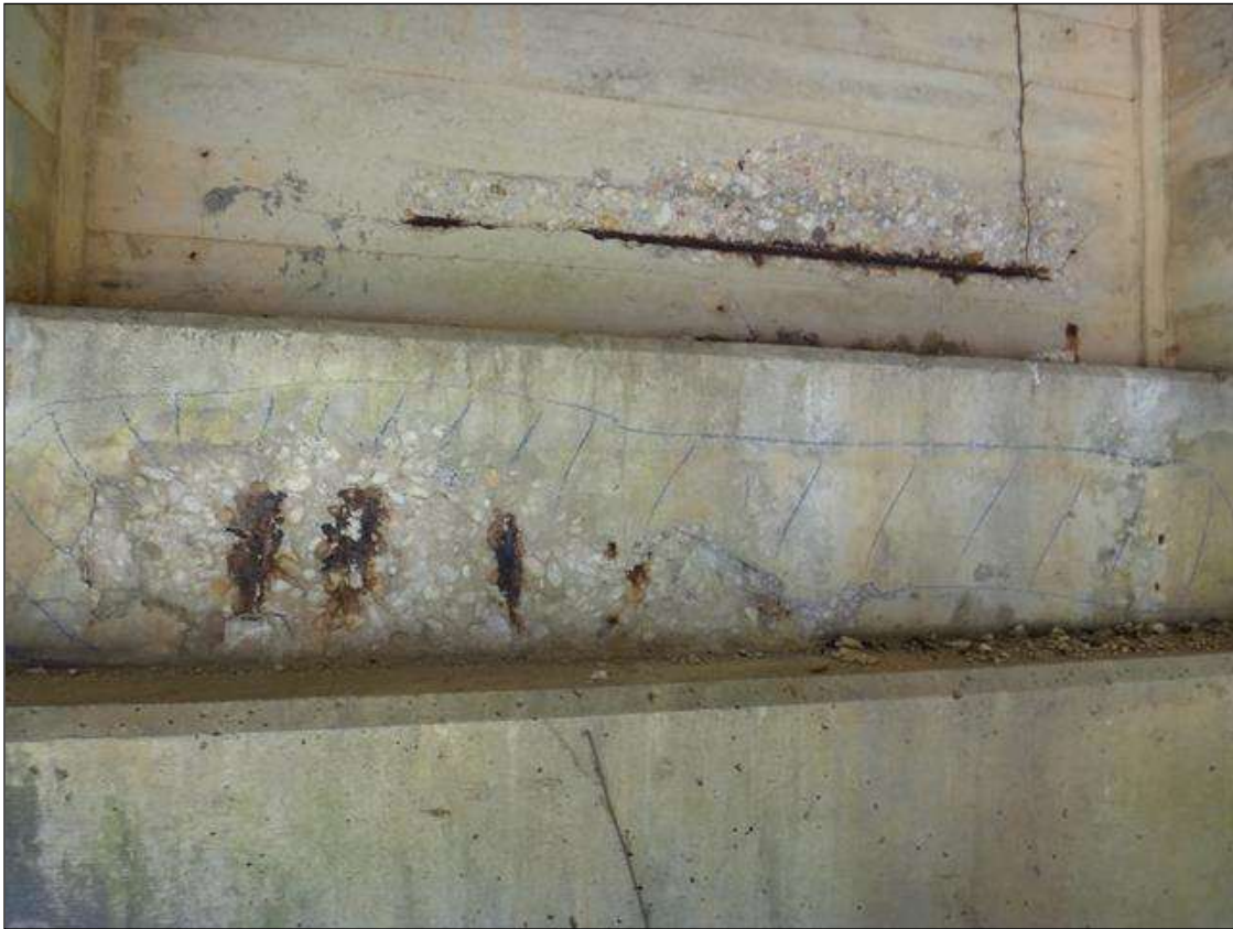
(PM) BENT 2 CAP WEST FACE AT BAY 2, SPALL (4FT X 12IN X 2IN) WITH EXPOSED RUSTED REBAR, SECTION LOSS (NO MEASURABLE LOSS), DELAMINATION (6-1/2FTX18IN)
