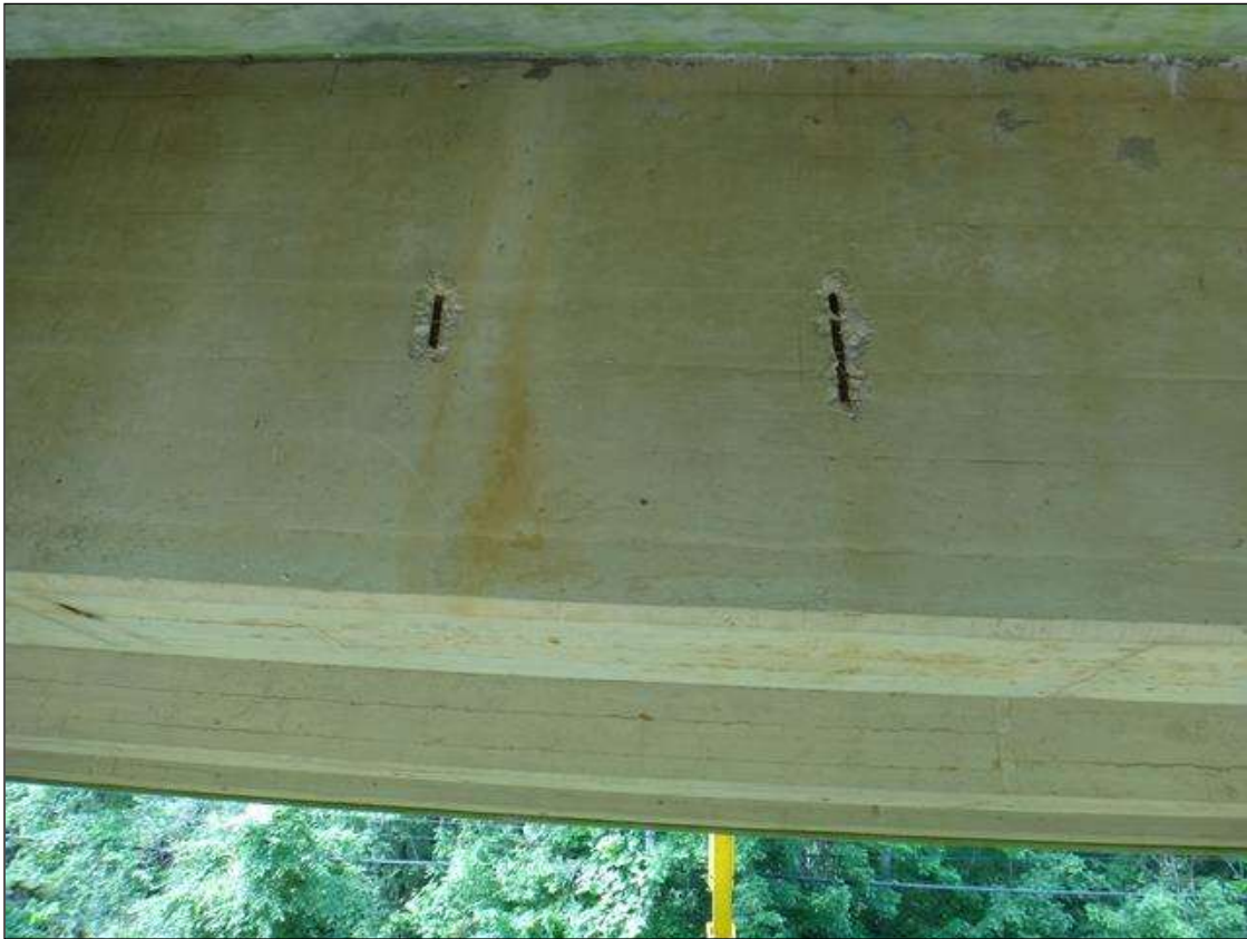
(PM) SPAN 4 BEAM 2 AT MIDSPAN, TWO (2) SPALLS (10IN X 3IN X 1IN DEEP) WITH EXPOSED RUSTED REBAR
