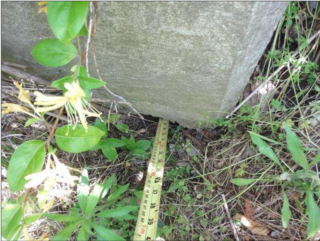
END BENT 2 CAP AT SOUTH END, EROSION WITH UNDERMINING (2FT X 1FT X 28IN)
