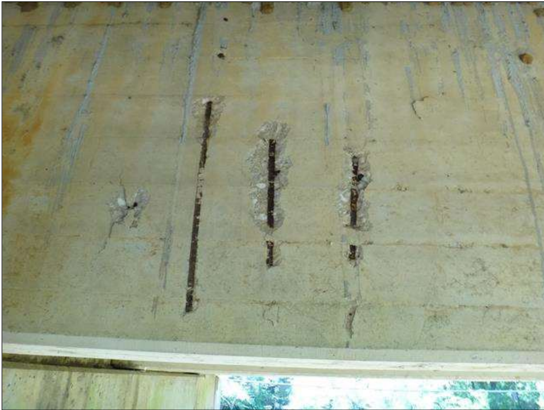
(PM) SPAN 8 BEAM 2 AT 6FT FROM BENT 8, MULTIPLE SPALLS (UP TO 2FT X 5IN X 1IN DEEP) WITH EXPOSED RUSTED REBAR
