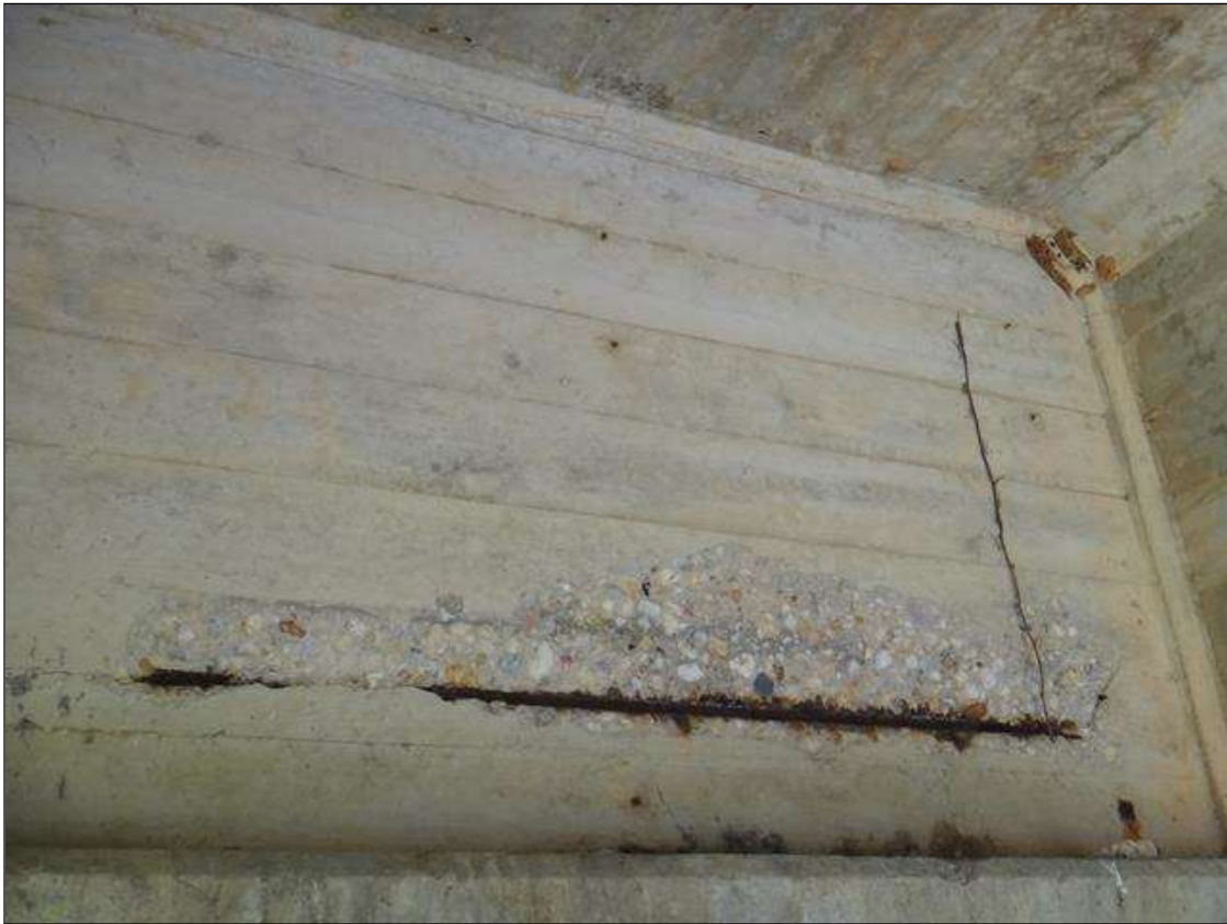
SPAN 2 BENT 2 BACKWALL AT BAY 2, SPALL (14IN X 6IN X 2IN DEEP) WITH EXPOSED RUSTED REBAR
