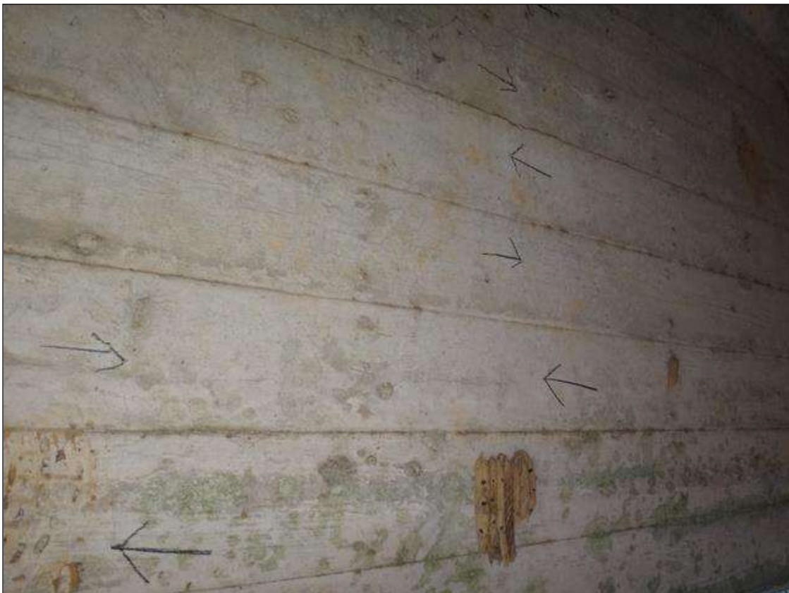
SPAN 10 BEAM 1 SOUTH FACE AT 10FT FROM END BENT 2, TWO (2) VERTICAL CRACKS (3FT X HAIRLINE)
