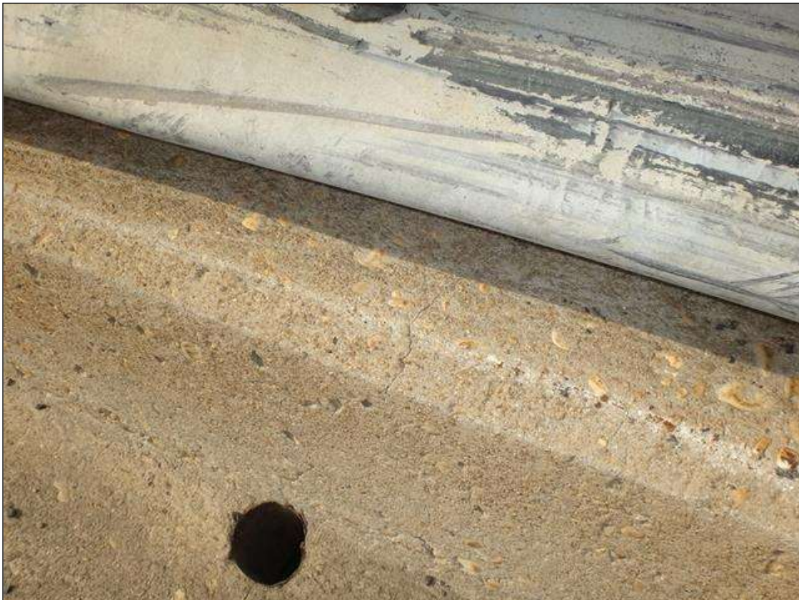
SPAN 1 SOUTH RAIL PARAPET AT 25FT FROM END BENT 1, TRANSVERSE CRACK (2FT X HAIRLINE)
