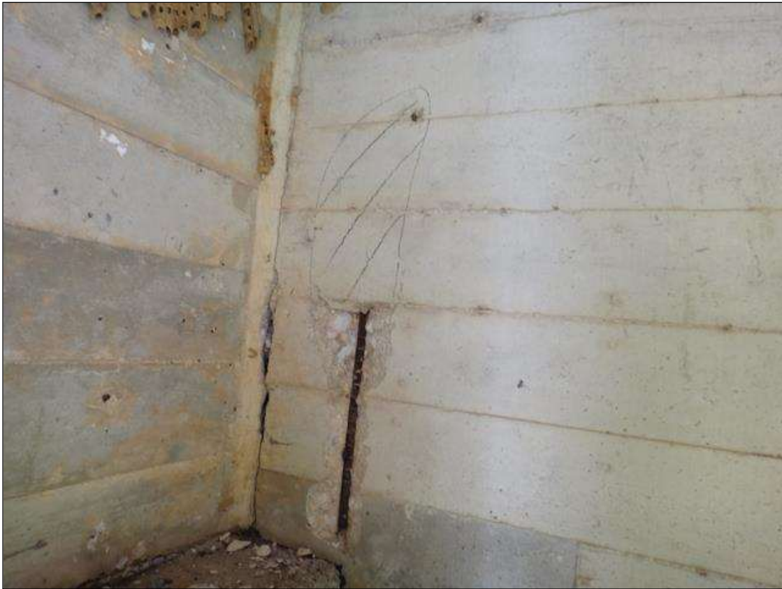
(PM) SPAN 9 BEAM 2 AT BENT 8, SPALL (16IN X 6IN X 1-1/2IN DEEP) WITH EXPOSED RUSTED REBAR, SECTION LOSS (NO MEASURABLE LOSS), ADJACENT DELAMINATION
