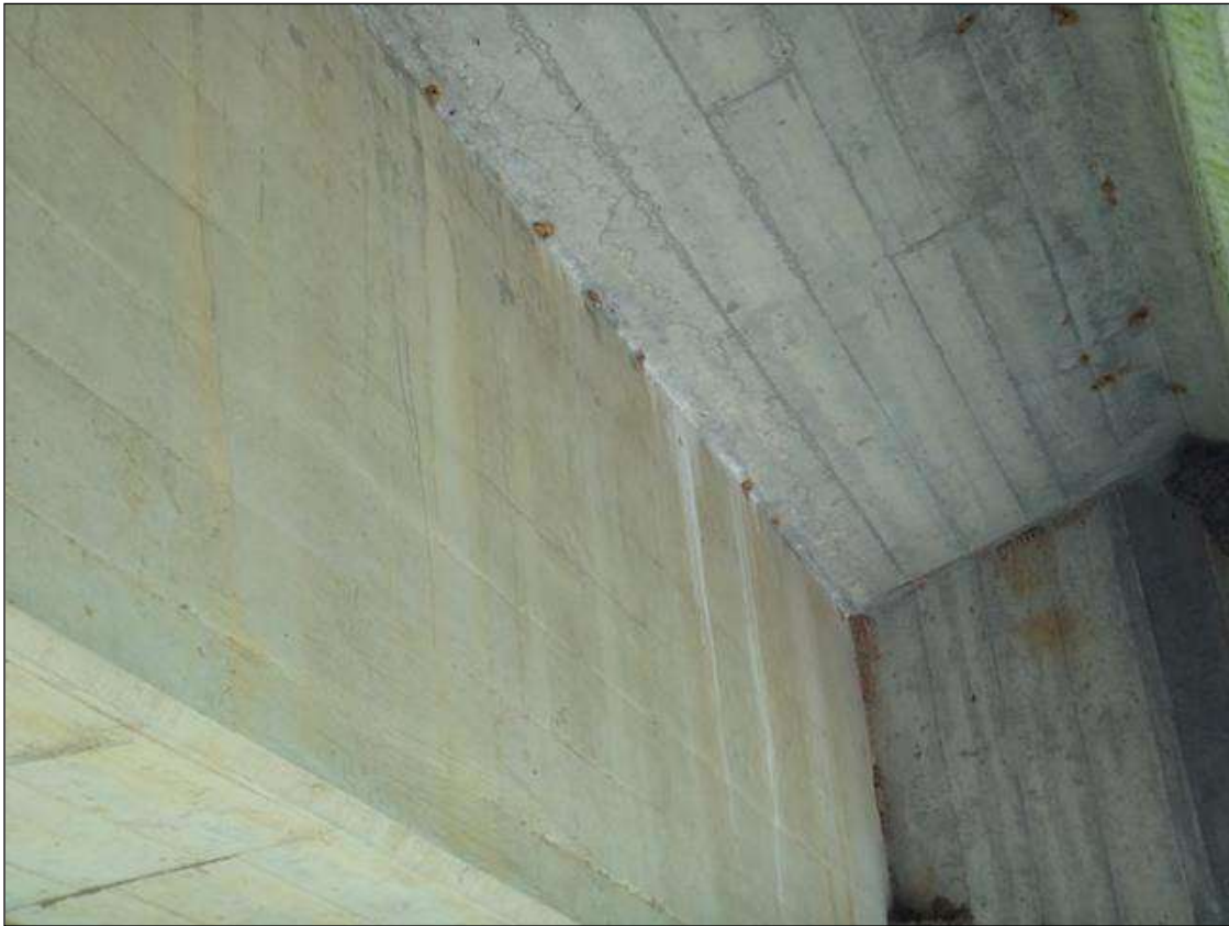
SPAN 4 UNDERSIDE OF DECK AT BAY 1, EFFLORESCENCE ALONG BENT 2 (ALL SPANS SIMILAR)
