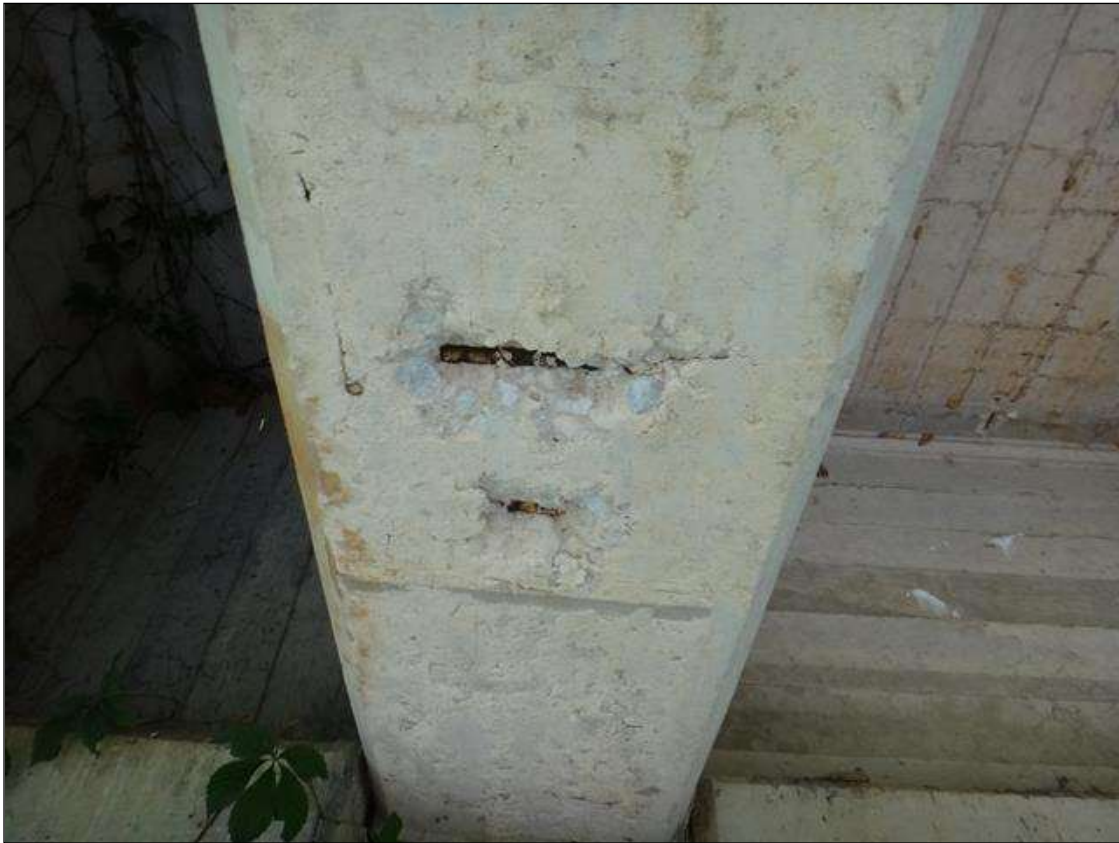
(PM) SPAN 9 BEAM 2 AT BENT 9, TWO (2) SPALLS (5IN DIAMETER X 1IN DEEP) WITH EXPOSED RUSTED REBAR
