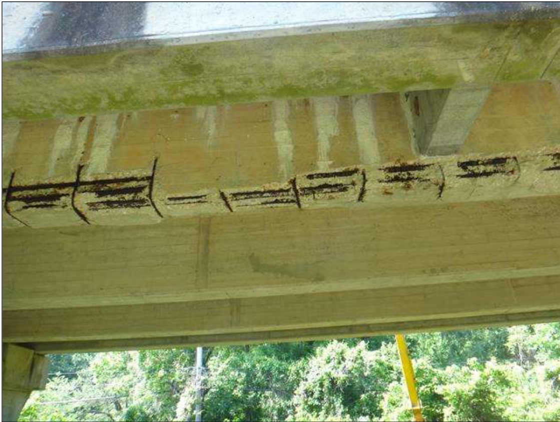
(PM) SPAN 6 BEAM 2 AT MIDSPAN, SPALL (26FT X 20IN X 2IN) WITH EXPOSED RUSTED REBAR, SECTION LOSS ON PRIMARY (NO MEASURABLE LOSS) AND SECONDARY (100%)
