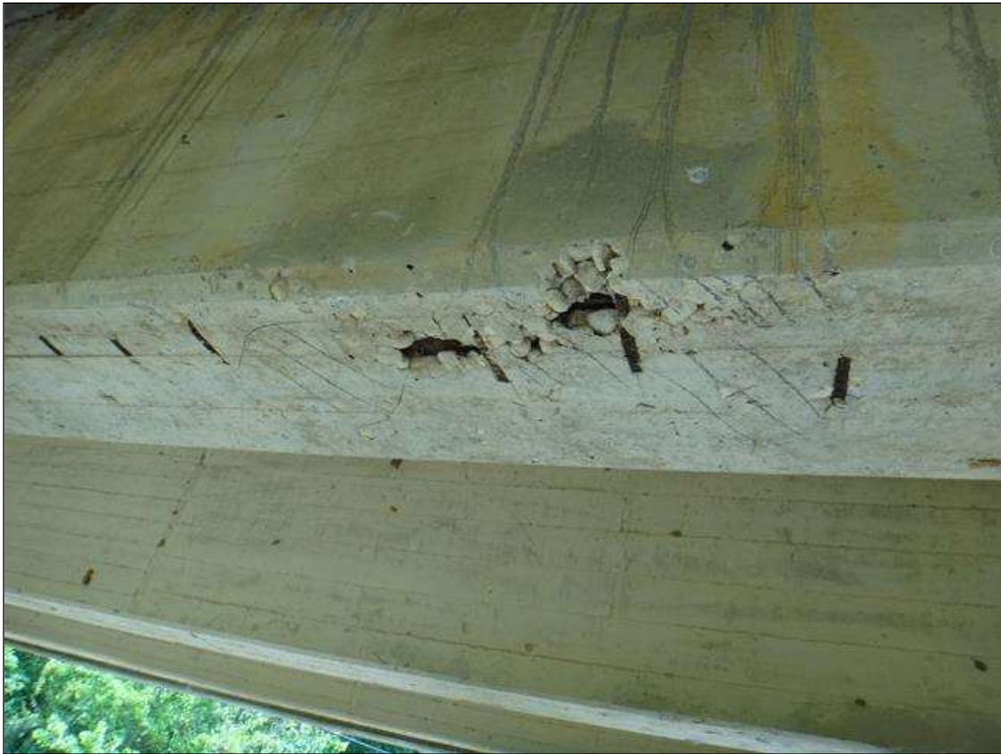
(PM) SPAN 9 BEAM 2 AT 5FT FROM BENT 8, SPALL (2FT X5INX 2IN) WITH EXPOSED RUSTED REBAR, HONEYCOMB, AND DELAMINATION, SECTION LOSS (NO MEASURABLE LOSS)
