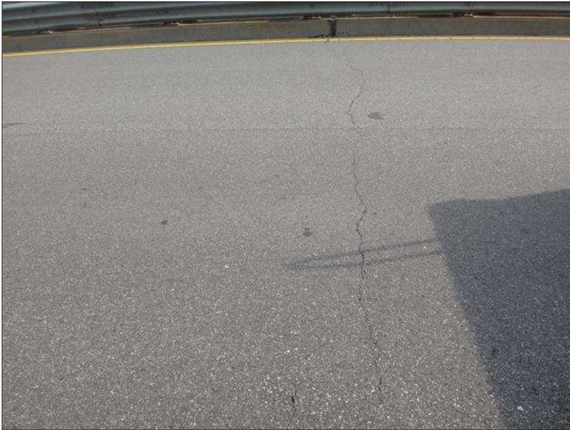
ASPHALT WEARING SURFACE OVER BENT 1, TRANSVERSE CRACK (FULL WIDTH X UP TO 1/4IN)
