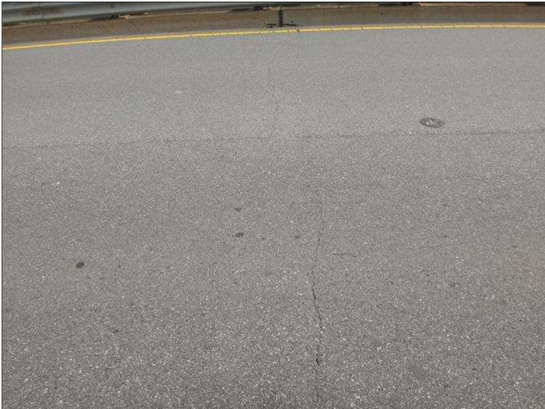
ASPHALT WEARING SURFACE OVER BENT 7, TWO (2) TRANSVERSE CRACKS (12FT X 1/8IN)
