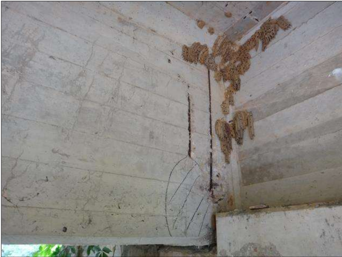
(PM) SPAN 9 BEAM 2 AT BENT 9, TWO (2) SPALLS (UP TO 40IN X 8IN X 1-1/2IN) WITH EXPOSED RUSTED REBAR, SECTION LOSS (NO MEASURABLE LOSS), DELAMINATION
