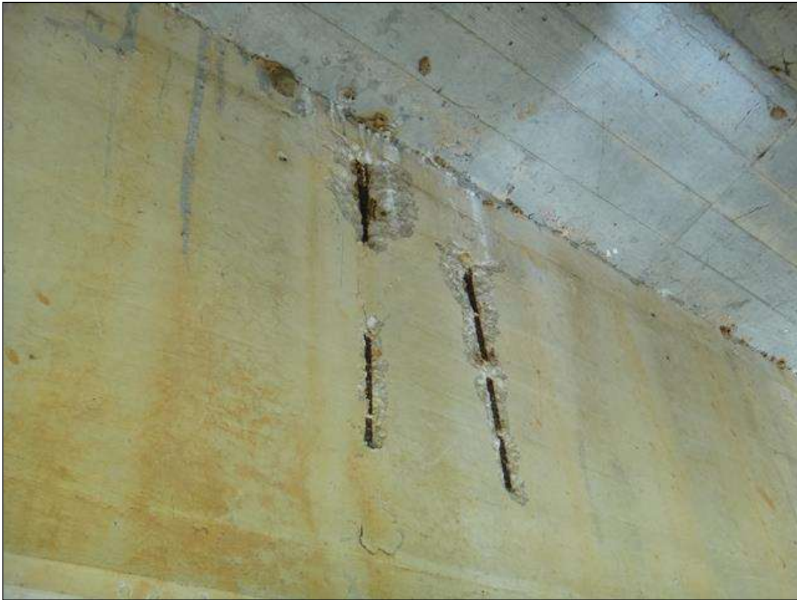
(PM) SPAN 9 BEAM 4 AT 12FT FROM BENT 8, MULTIPLE SPALLS/DELAMINATIONS (UP TO 26IN X 5IN X 1IN DEEP) WITH EXPOSED RUSTED REBAR
