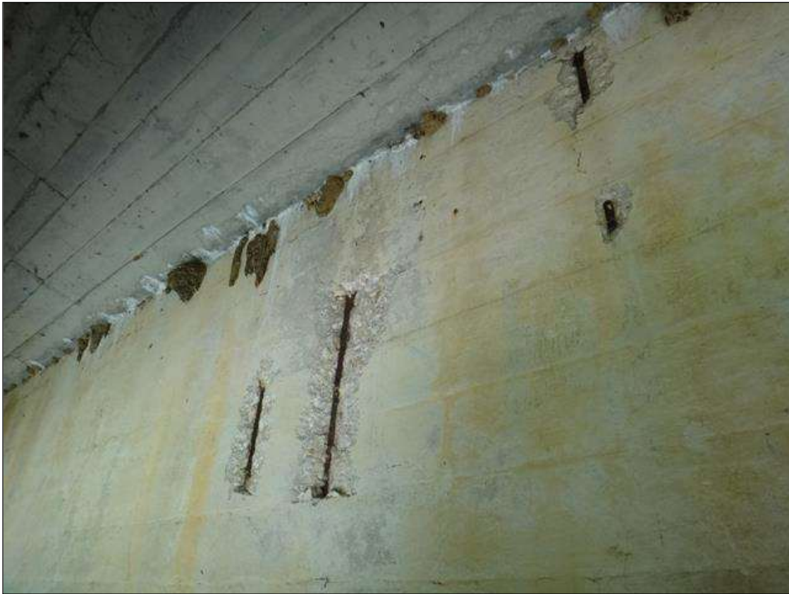
(PM) SPAN 7 BEAM 2 AT 12FT FROM BENT 6, MULTIPLE SPALLS (UP TO 18IN X 12IN X 1IN) WITH EXPOSED RUSTED REBAR AND SECTION LOSS, ADJACENT DELAMINATION
