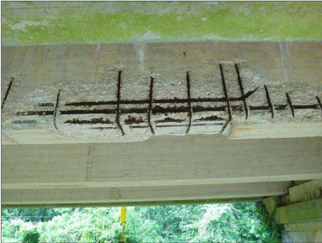
(PM) SPAN 5 BEAM 2 AT WEST HALF, SPALL (15FT X 2FT X 3IN DEEP) WITH EXPOSED RUSTED REBAR, SECTION LOSS (NO MEASURABLE LOSS), DEBONDED REBAR
