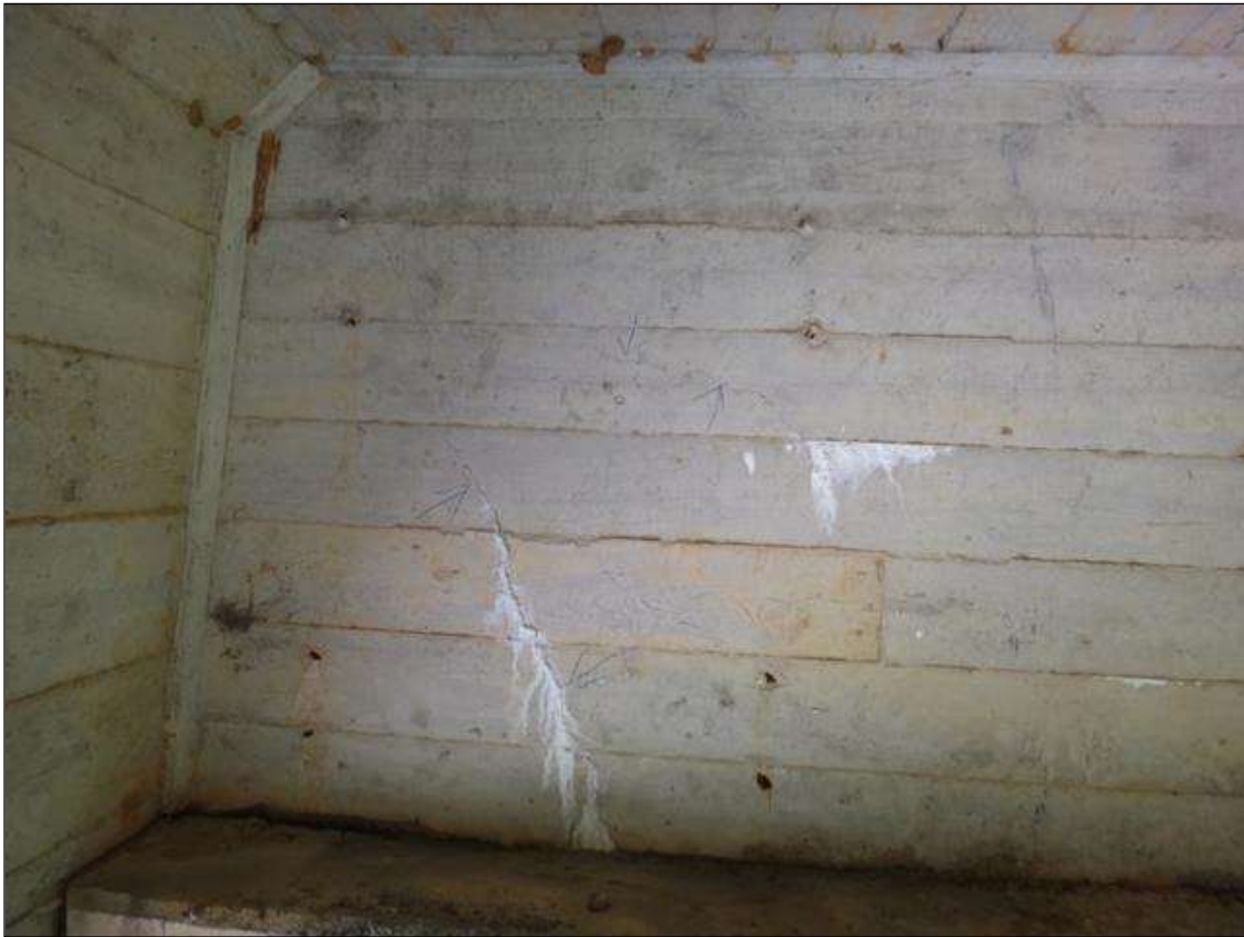
SPAN 5 BENT 5 BACKWALL AT BAY 3, TWO (2) DIAGONAL CRACKS (UP TO FULL HEIGHT X HAIRLINE) WITH EFFLORESCENCE
