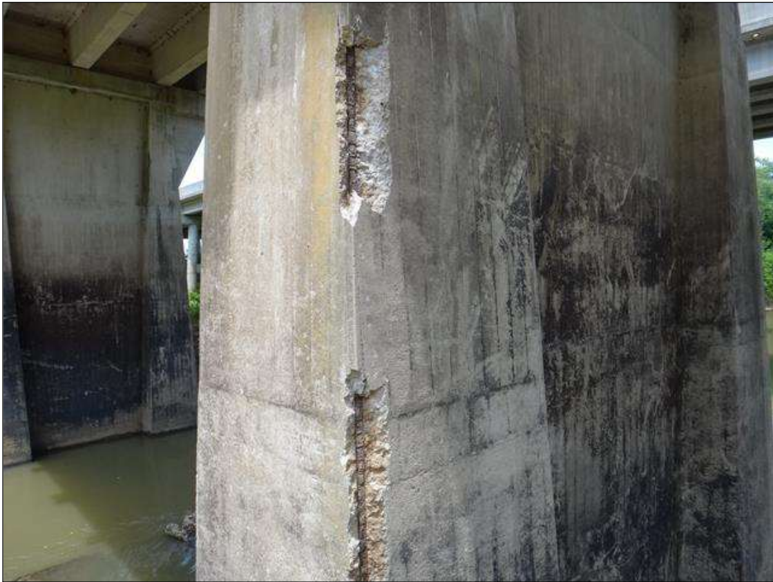
(PM) BENT 8 COLUMN 2 SOUTHEAST CORNER AT 10FT ABOVE WATERLINE, TWO (2) SPALLS (UP TO 4FT X 6IN X 2IN) WITH EXPOSED RUSTED REBAR AND SECTION LOSS
