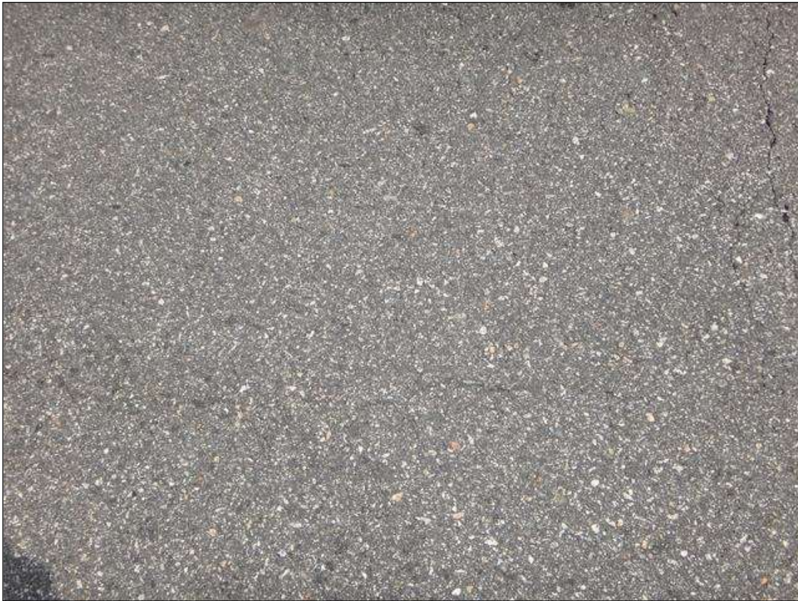
SPAN 10 ASPHALT WEARING SURFACE RIGHT LANE AT END BENT 2, LONGITUDINAL CRACK (3FT X 1/16IN)
