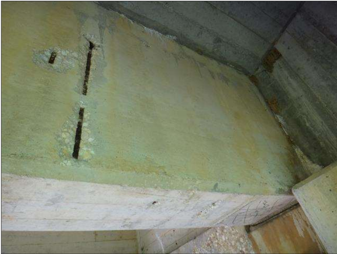
(PM) SPAN 5 BEAM 4 AT BENT 5, MULTIPLE SPALLS (UP TO 24IN X 4IN X 1IN DEEP) WITH EXPOSED RUSTED REBAR AND SECTION LOSS, DELAMINATION (18IN X 18IN)
