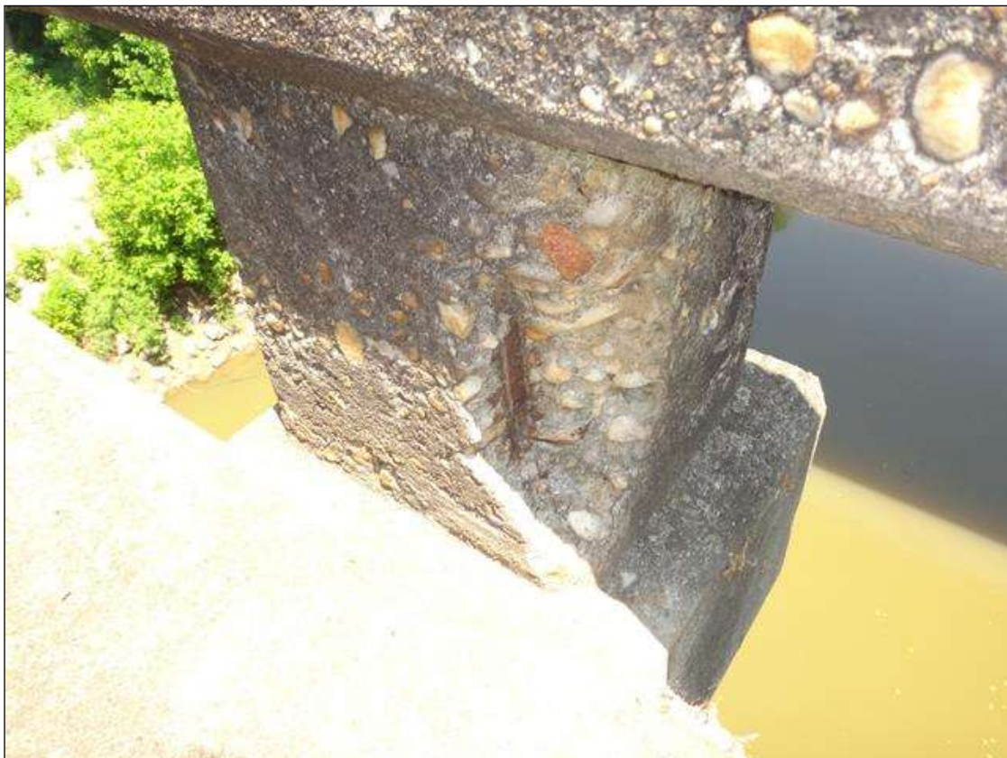
SPAN 9 NORTH RAIL POST AT 10FT FROM BENT 8, SPALL (8IN X 4IN X 1-1/2IN DEEP) WITH EXPOSED RUSTED REBAR
