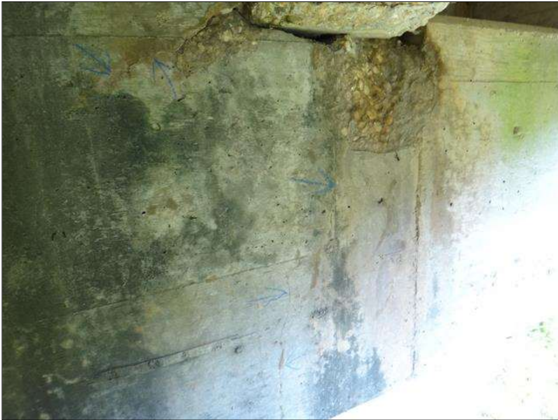
BENT 1 CAP EAST FACE BELOW BEAM 2, TWO (2) SPALLS (UP TO 15IN X 11IN X 2IN DEEP) WITH VERTICAL CRACKS (UP TO FULL HEIGHT X HAIRLINE)
