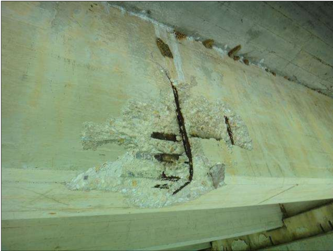
(PM) SPAN 7 BEAM 2 AT 12FT FROM BENT 6, SPALL (3FT X 3FT X 3IN DEEP) WITH EXPOSED RUSTED REBAR, SECTION LOSS (NO MEASURABLE LOSS)
