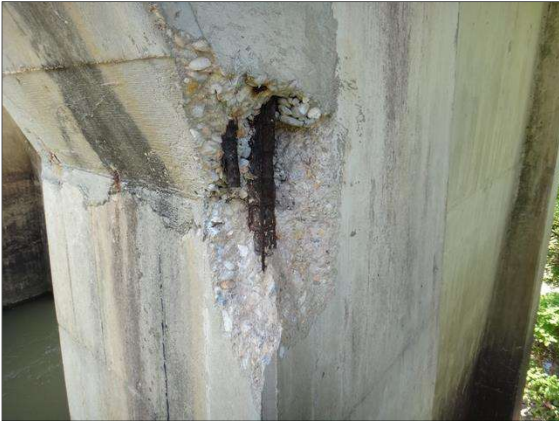
(PM) BENT 7 COLUMN 1 NORTHWEST CORNER AT HAUNCH, SPALL (24IN X 8IN X 4IN) WITH EXPOSED RUSTED REBAR, SECTION LOSS (NO MEASURABLE LOSS)
