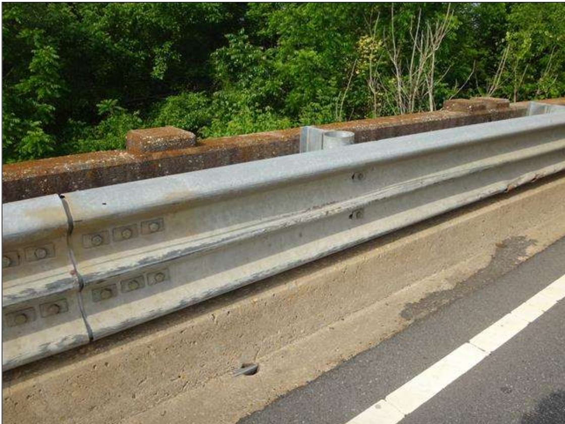
SPAN 2 SOUTH RAIL NEAR MIDSPAN, IMPACT DAMAGE/SCRAPES (20FT)
