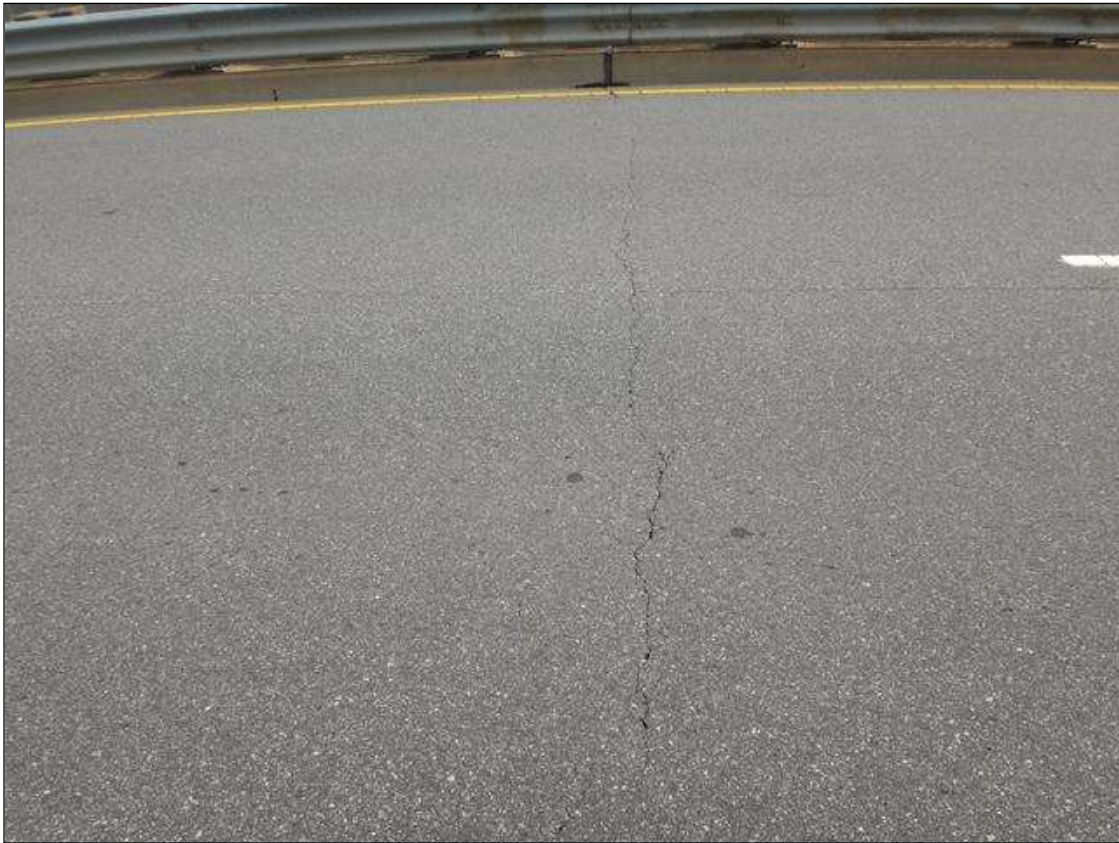
ASPHALT WEARING SURFACE OVER BENT 8, TRANSVERSE CRACK (FULL WIDTH X 1/8IN)
