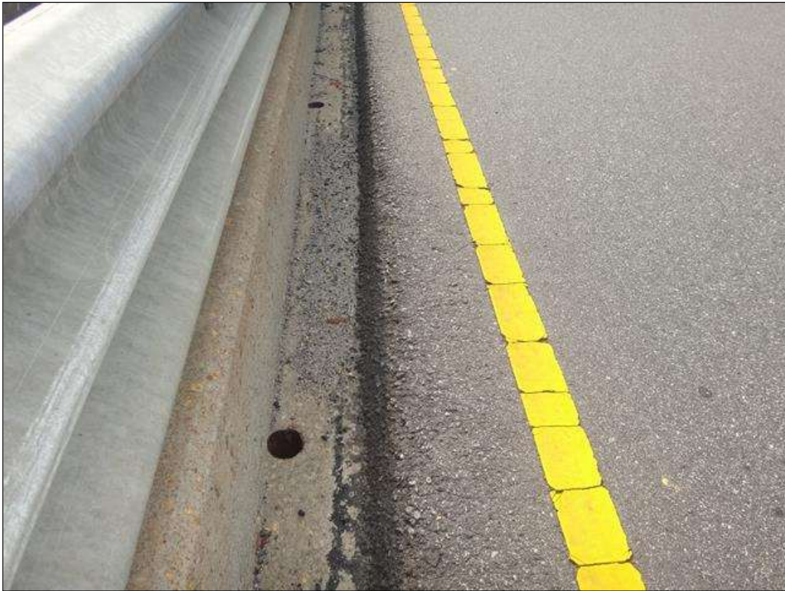
NORTH CURB, DROPOFF (UP TO 4IN) FROM ASPHALT WEARING SURFACE
