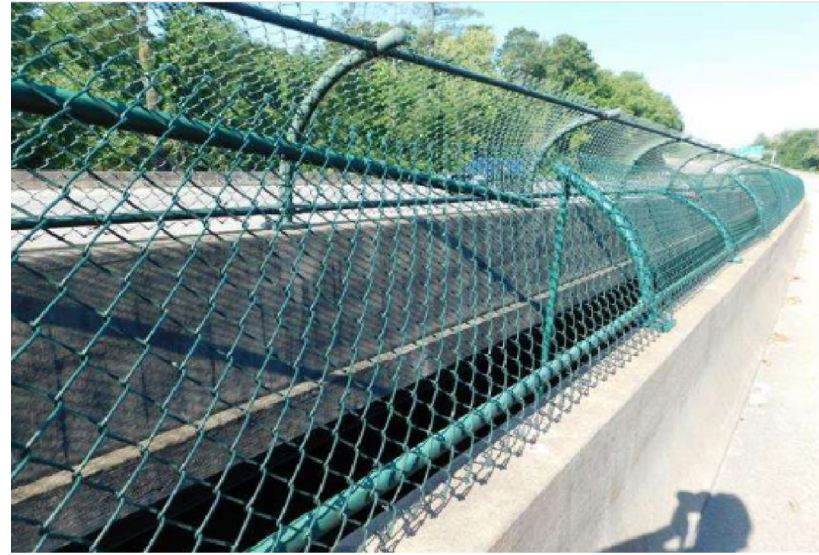
EXISTING FENCE DAMAGE
