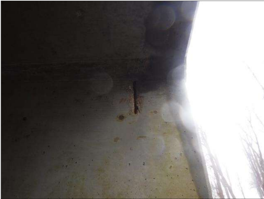
Barrel 2 Section 1: SPALL WITH EXPOSED REBAR NEAR WEST END ON INTERIOR WALL 1' LONG X 3" WIDE X 1/2" DEEP
