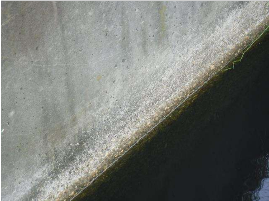
COARSE AGGREGATE EXPOSED ON WINGS
