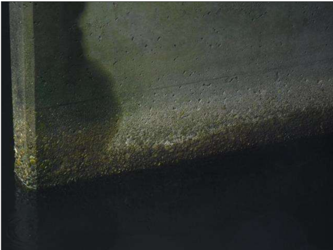
COARSE AGGREGATE EXPOSED ON INTERIOR WALLS
