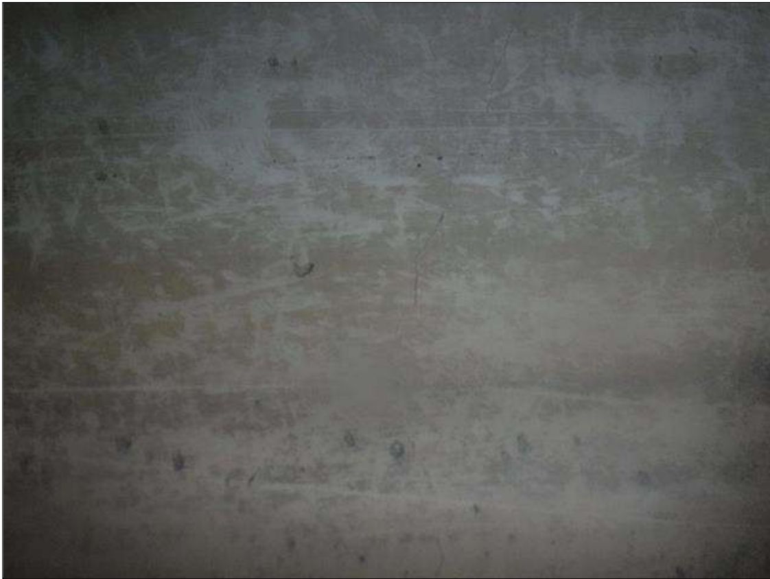
Barrel 3 Section 1: 2' H/L VERTICAL CRACKS IN INTERIOR WALL
