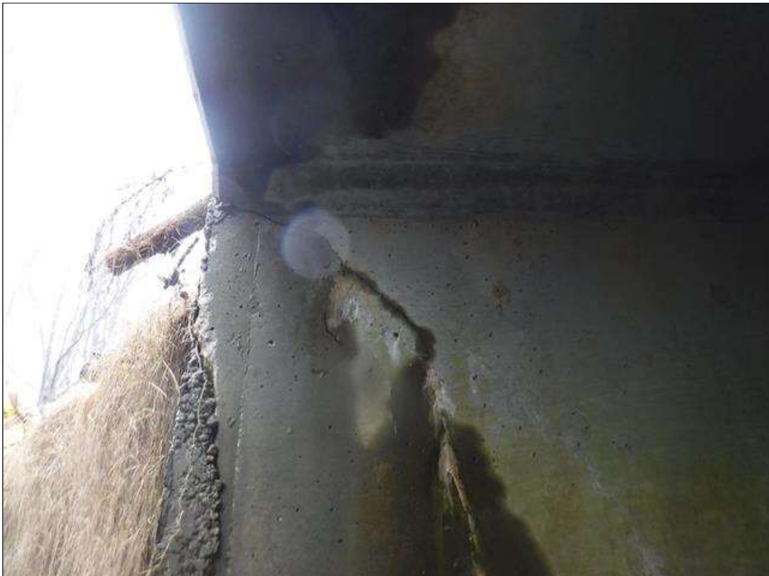
Barrel 3 Section 1: DIAGONAL CRACKING WITH EFFLO. TO 1/16" ON EXTERIOR WALL AT WEST END
