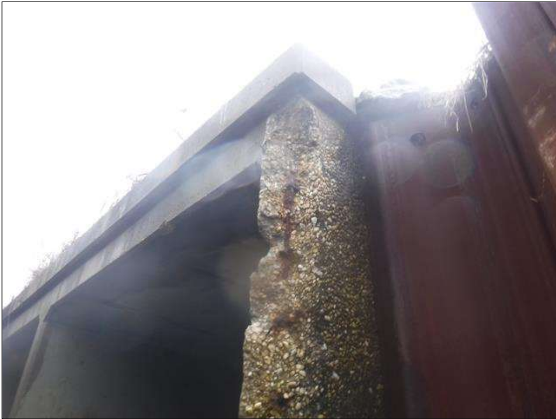
Barrel 1 Section 1: DAMAGE FULL HEIGHT AT UPSTREAM END OF EXTERIOR WALL FROM WING BEING TORN OFF DURING STORM FLOODING.
