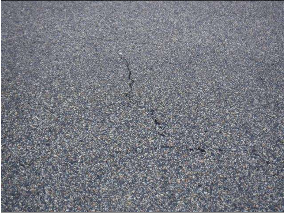
ROADWAY CRACKING IN SOUTH BOUND LANES
