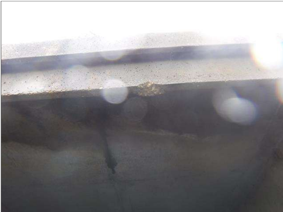
Barrel 1 Section 1: SPALL AT WEST END ON TOP SLAB 4" DIAMETER X 1.5" DEEP
