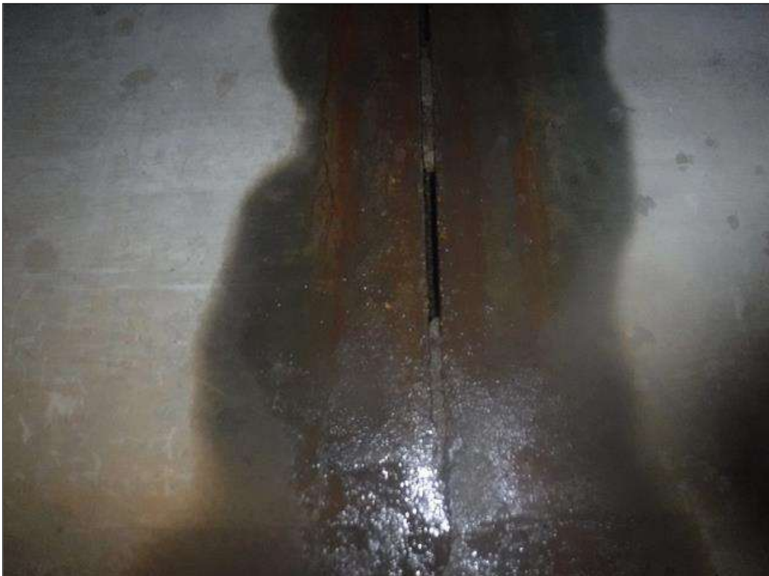
Barrel 3 Section 1: CONSTRUCTION JOINT OPEN TO 1/2"
