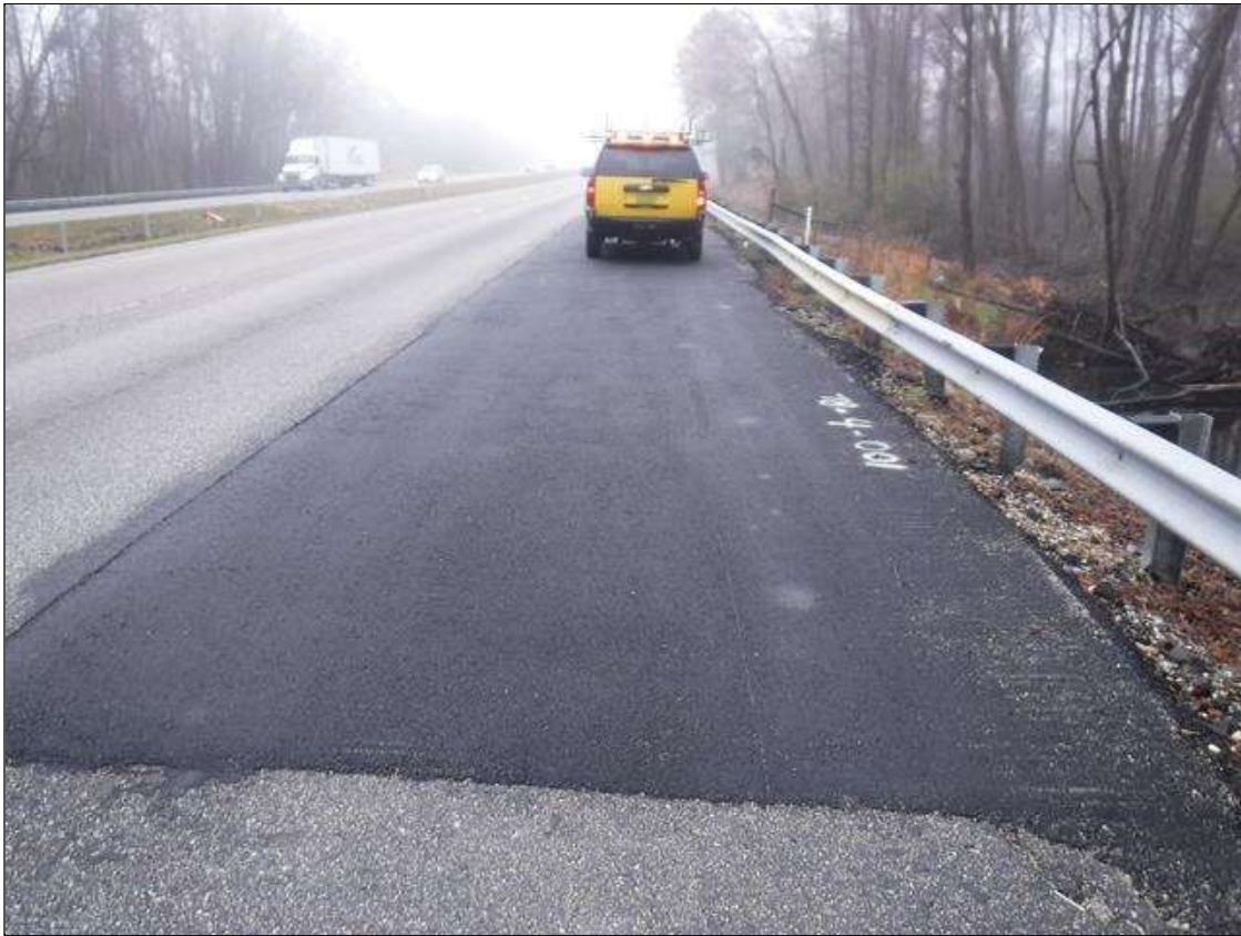
PATCHED AREA WEST SHOULDER
