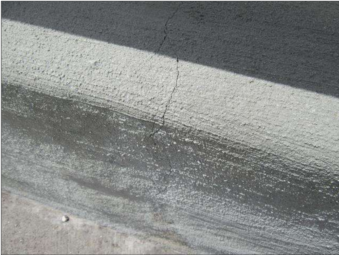
Span 2 Left Bridge Rail: HAIRLINE TRANSVERSE AND VERTICAL CRACKS AT 4-6 FT. SPACING
