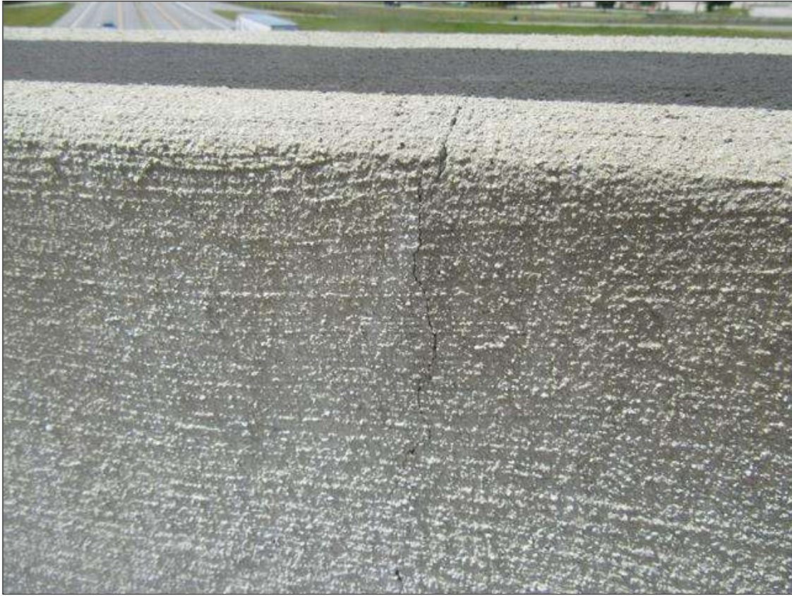
Span 1 Left Bridge Rail: HAIRLINE TRANSVERSE AND VERTICAL CRACKS AT 4-6 FT. SPACING
