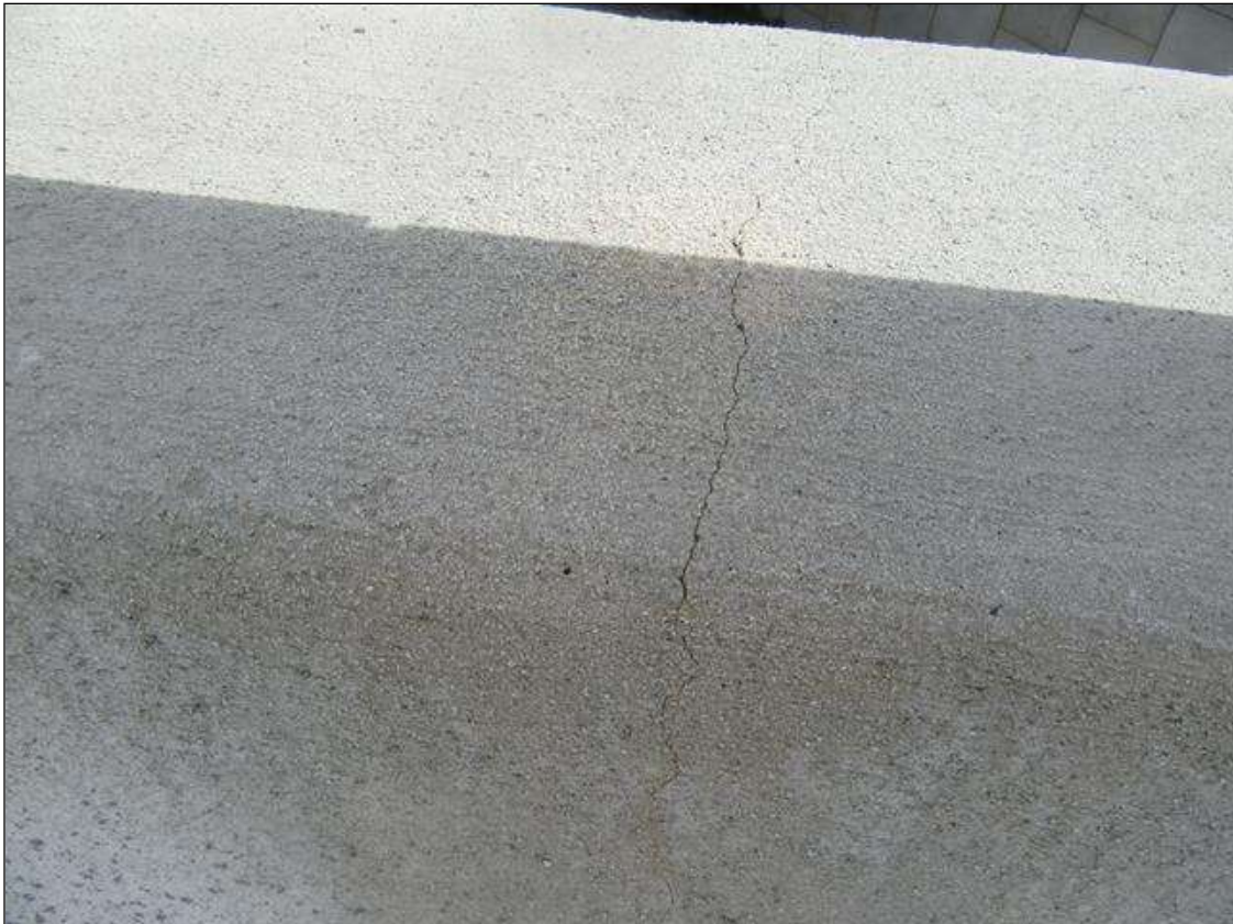
Span 1 Right Bridge Rail: HAIRLINE TRANSVERSE AND VERTICAL CRACKS AT 4-6 FT. SPACING
