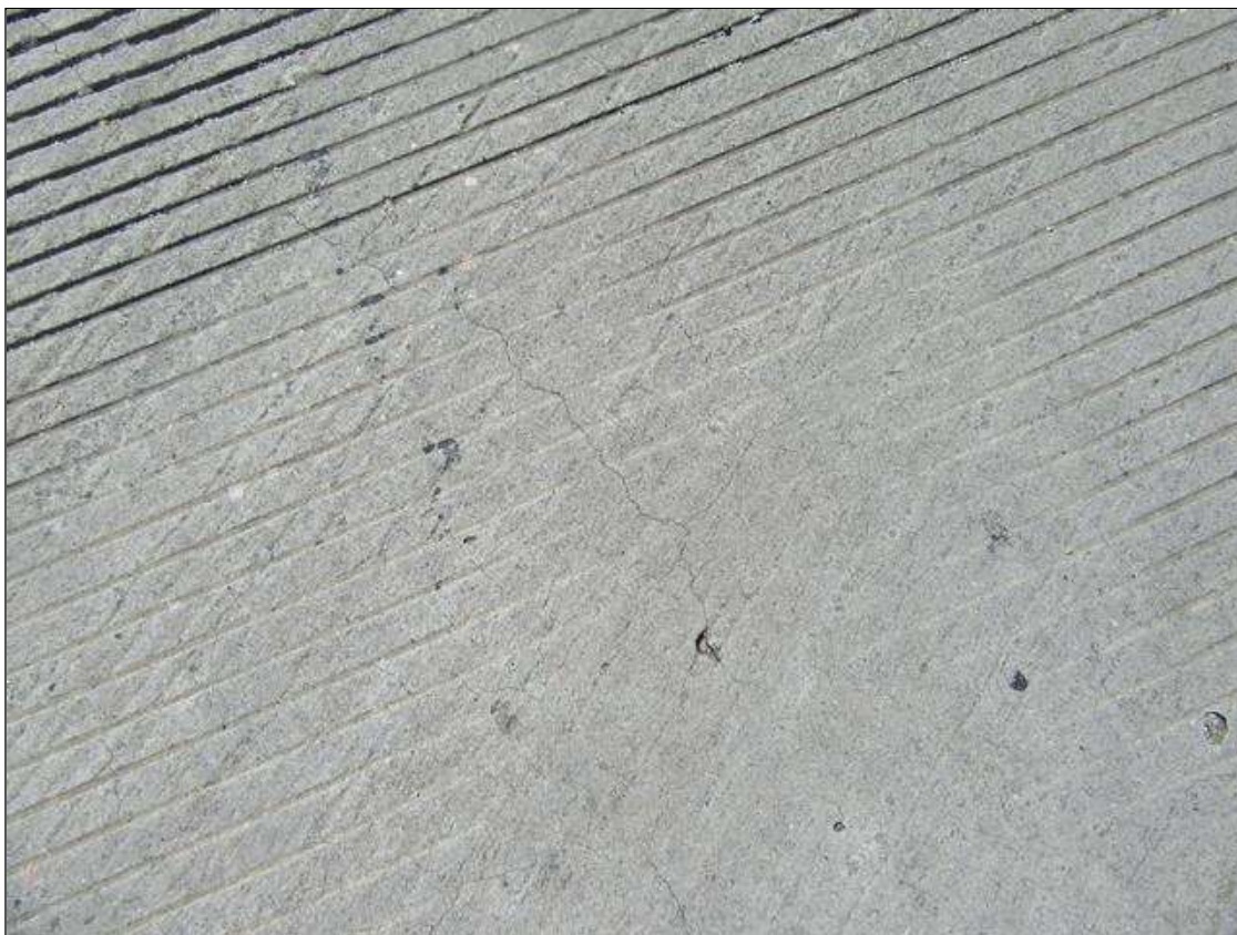
Approach 1: HAIRLINE LONGITUDINAL CRACKS AT END BENT 1 JOINT
