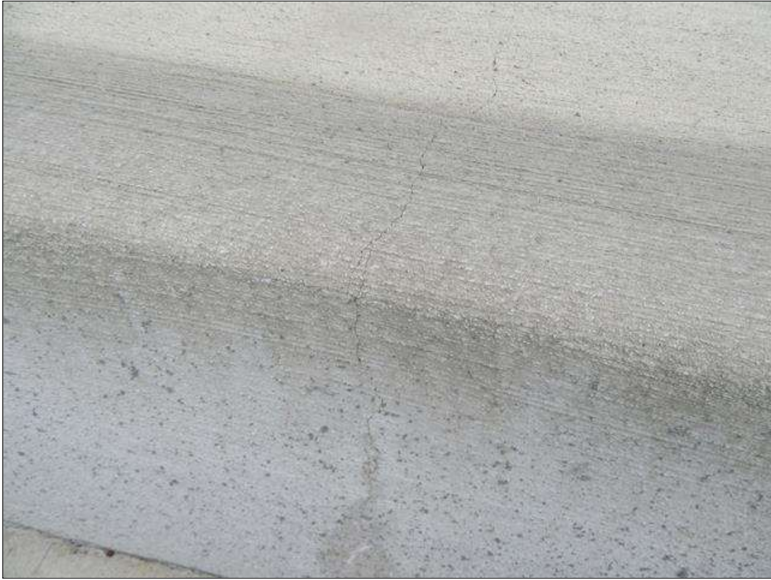
Span 2 Right Bridge Rail: HAIRLINE TRANSVERSE AND VERTICAL CRACKS AT 4-6 FT. SPACING
