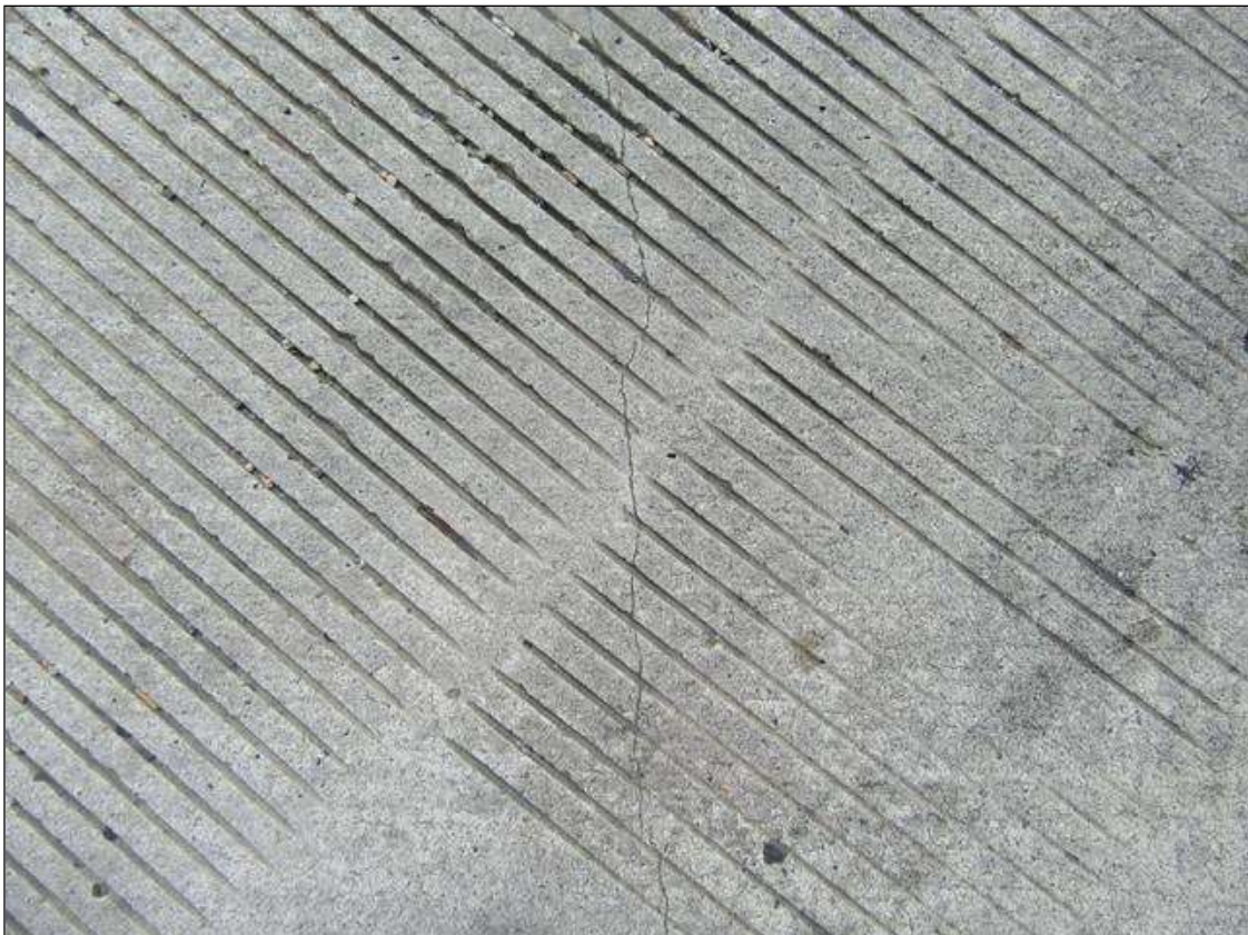
Span 2 Deck: 9- 2 FT. LONG X HAIRLINE LONGITUDINAL CRACKS AT END BENT 2 JOINT
