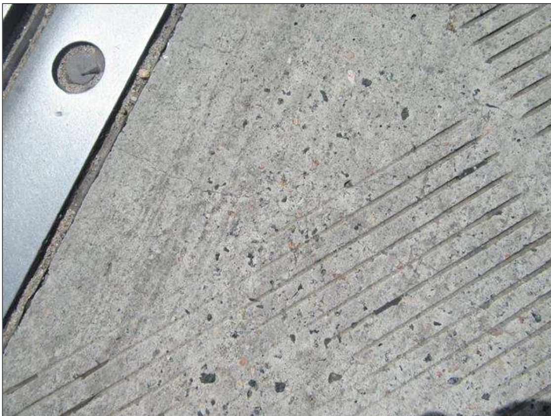
Span 1 Deck: 6 - 2 FT. LONG X HAIRLINE LONGITUDINAL CRACKS AT END BENT 1 JOINT
