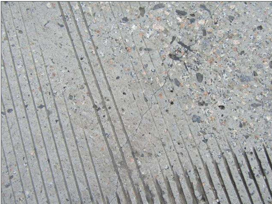
Approach 2: HAIRLINE LONGITUDINAL CRACKS AT END BENT 2 JOINT
