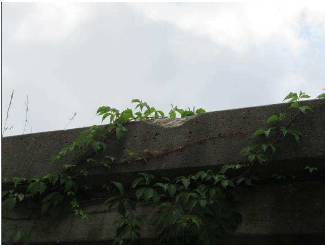
WEST HEADWALL SPALL 8" LONG X 3" HIGH X 2" DEEP OVER BARREL 2
