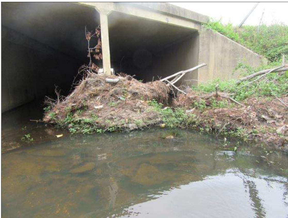
DRIFT AT EAST END INTERIOR WALL 20 HOURS.
