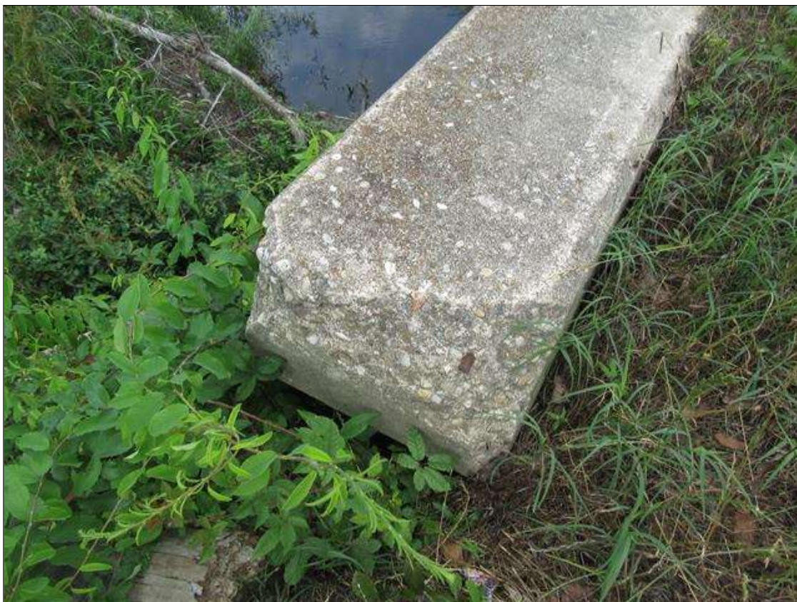
EAST HEADWALL SPALL 16" LONG X 8" WIDE X 6" DEEP AT NORTHEAST CORNER
