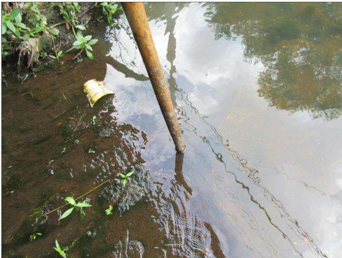
6" OF VERTICAL SCOUR AT EAST END OF BARREL 1
