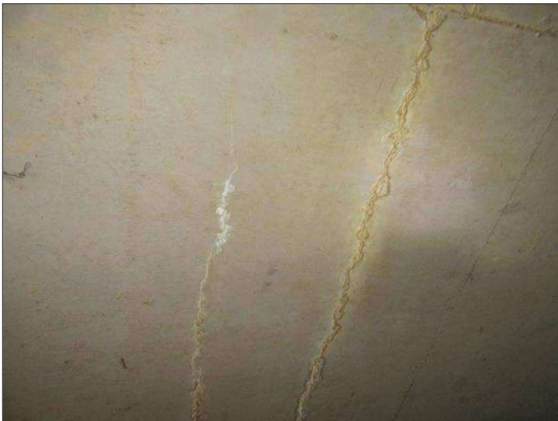
Barrel 2 Section 1: 10 - 10 FT. LONG HAIRLINE LONGITUDINAL CRACKS WITH EFFLORESCENCE AT 5-20 FT. SPACING
