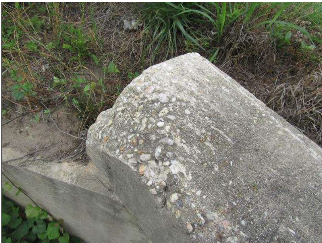
EAST HEADWALL SPALL 16" LONG X 12" WIDE X 8" DEEP AT SOUTHEAST CORNER
