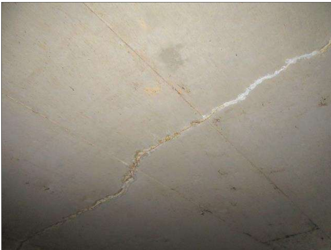
Barrel 1 Section 1: 2 - 10 FT. LONG X HAIRLINE LONGITUDINAL CRACKS WITH EFFLORESCENCE IN TOP SLAB AT 50 FT. FROM EAST END
