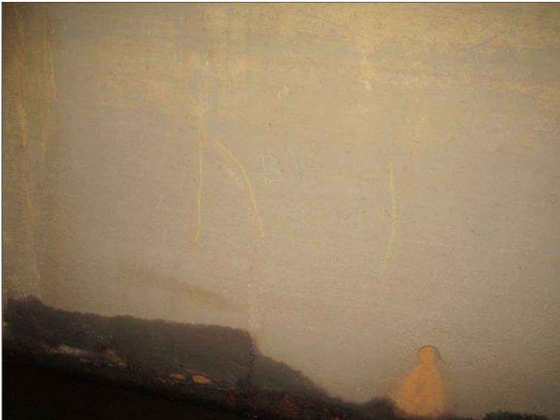
Barrel 1 Section 1: 3 - 5 FT. HIGH X HAIRLINE VERTICAL CRACKS AT 2 FT. SPACING IN SOUTH WALL 75' FROM EAST END
