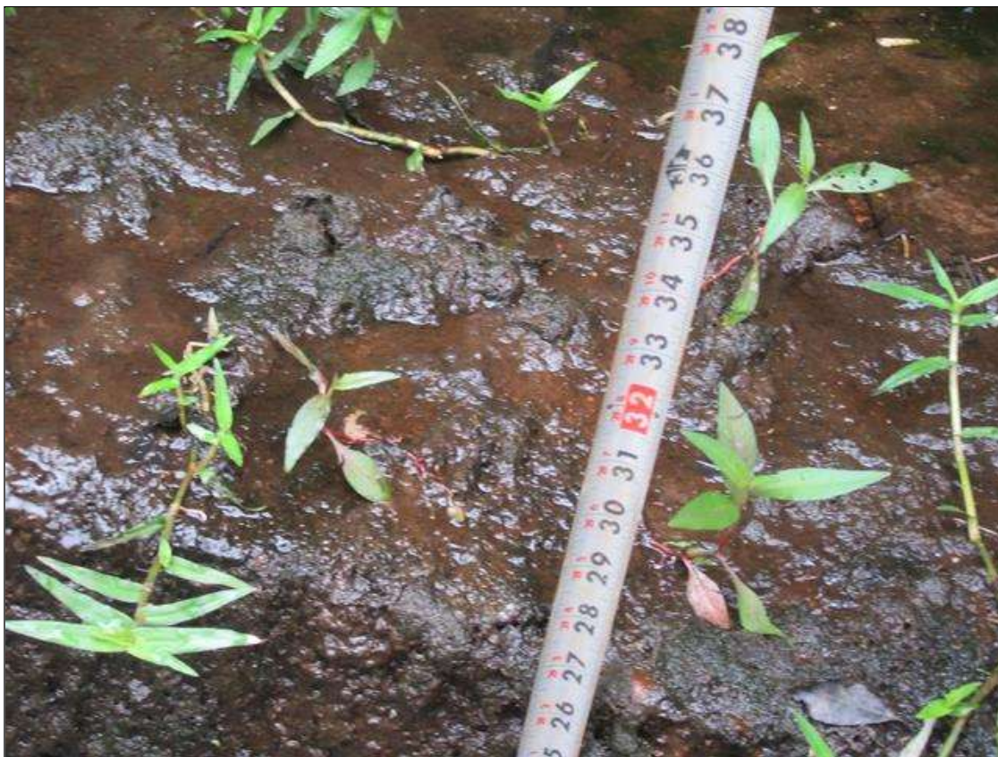
2.25 FT. VERTICAL SCOUR AT WEST OUTLET END OF BARRELS 1 AND 2 WITH NO UNDERMINING
