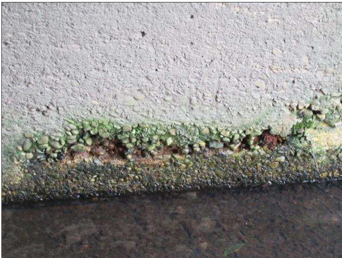
Barrel 1 Section 1: SPALL 2 FT. LONG X 2-3" HIGH X 1" DEEP IN BARREL 1 SOUTH WALL AT WEST END
