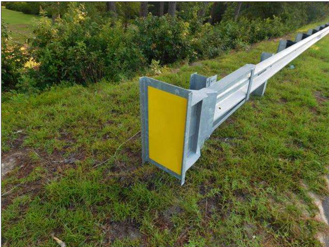
GUARDRAIL END TERMINAL
