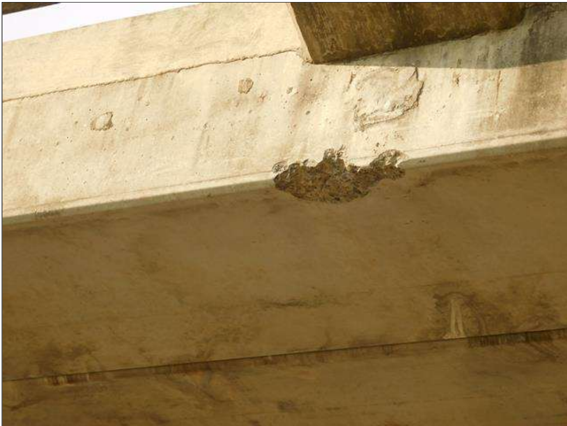
Span 2 Slab 1: OUTBOARD LOWER SIDE OF THE SLAB HAS PAST IMPACT DAMAGE, APPROX 1'L X UP TO 5"W X UP TO 2"D, CENTERED OVER THE RT SOUTHBOUND LANE
