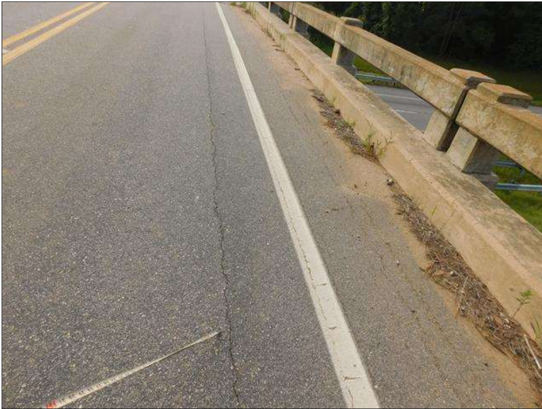
Span 2 Wearing Surface: LONGITUDINAL REFLECTIVE CRACKING UP TO .010 WIDE, RT LANE, LT SHOULDER AND RIGHT SHOULDER
