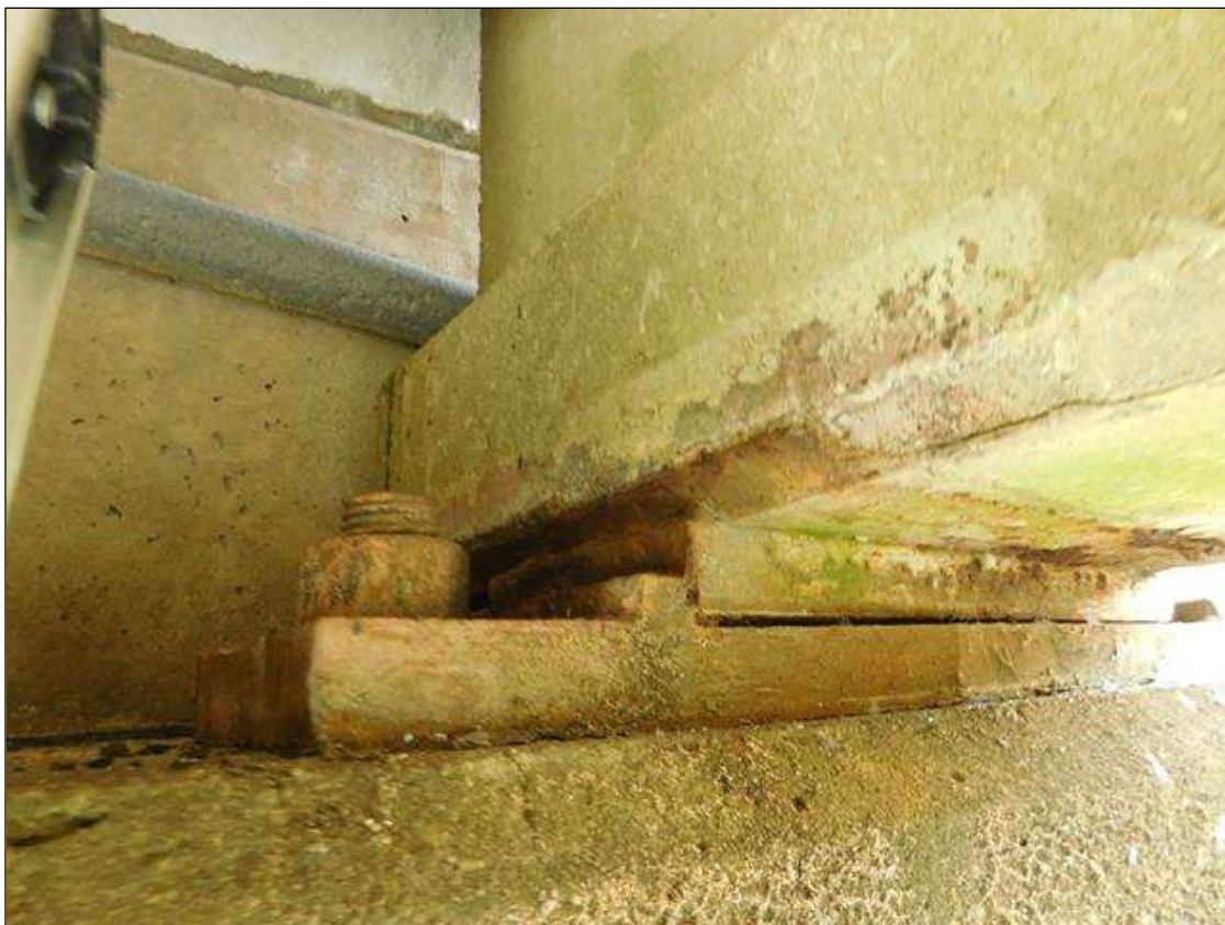
Span 4 Beam 1 Near Bearing: FRECKLED CORROSION
