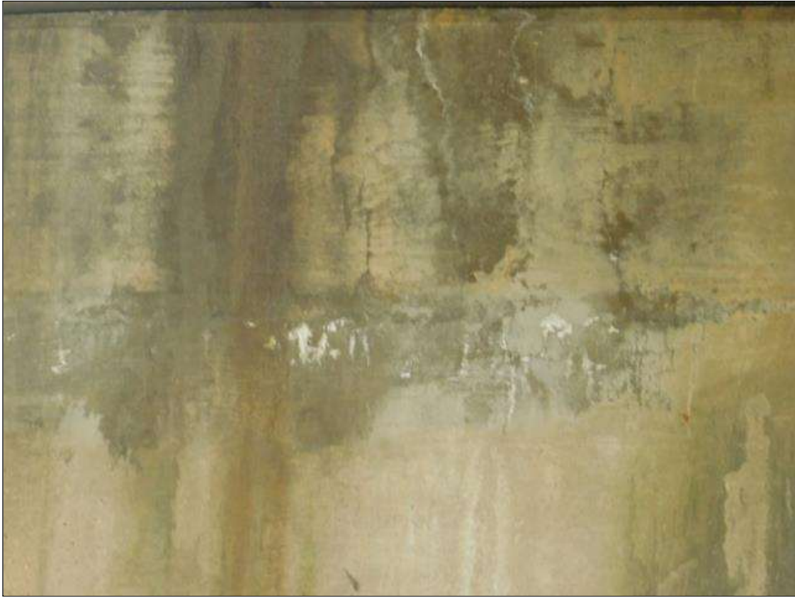
Bent 2 Cap 1: 1 Feet of longitudinal Cracking (RC and Other): Width .005 open on bottom face under slabs 4 and 5.
