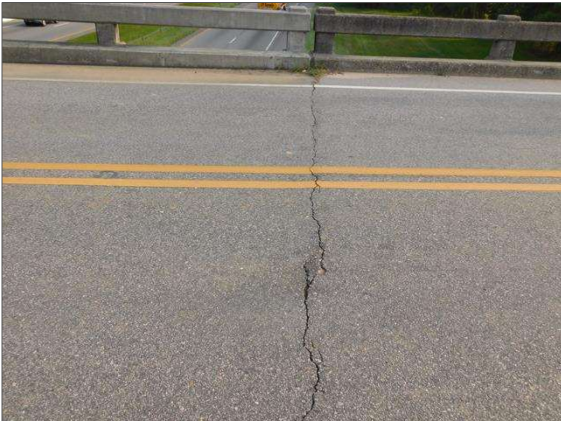
Span 3 Wearing Surface: OVER BENT 3, FULL WIDTH TRANSVERSE CRACKING UP TO .042 WIDE WITH IMPENDING POPOUTS
