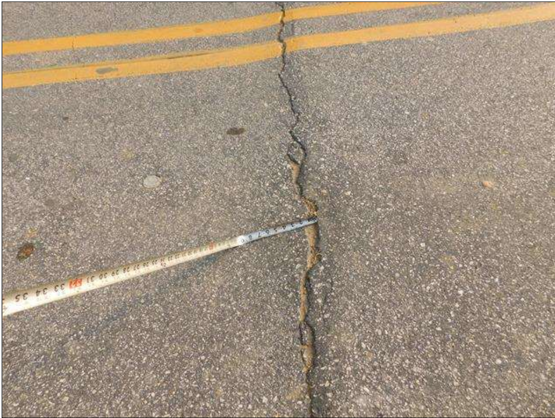
Span 1 Wearing Surface: UP TO .103 FT. WIDE TRANSVERSE CRACK OVER END BENT 1
