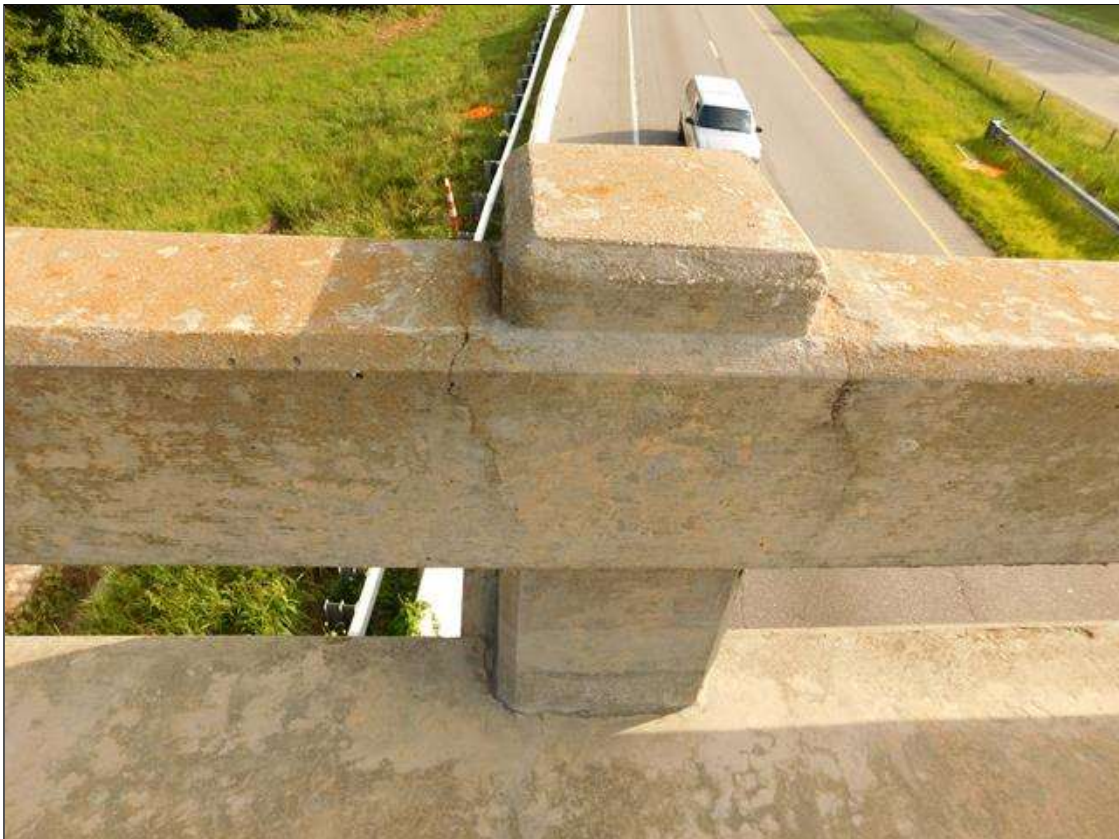
Span 2 Left Bridge Rail: 2 HAIRLINE VERTICAL CRACKS AT POST 2 AND 2 HAIRLINE VERTICAL CRACKS AT POST 8
