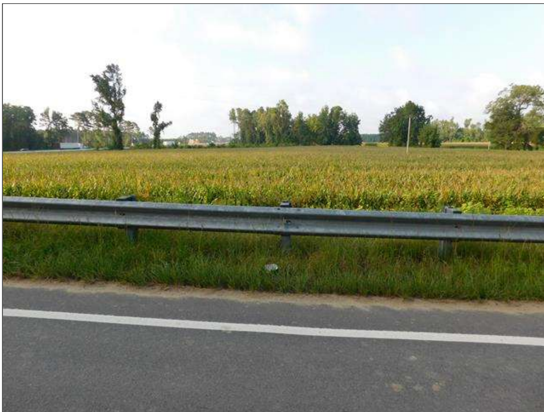
GUARDRAIL POST SPACING AT MID PORTION
