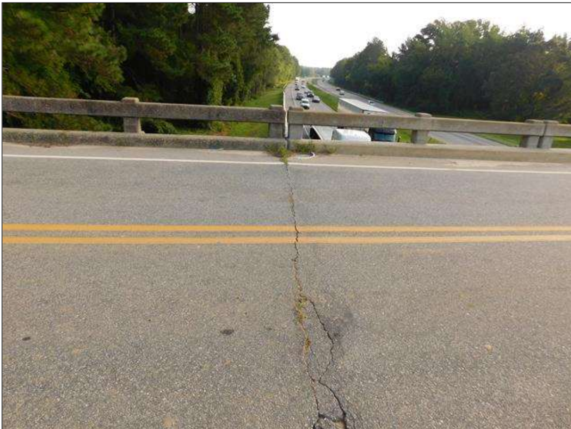
Span 1 Wearing Surface: .005 WIDE TRANSVERSE CRACK OVER BENT 1
