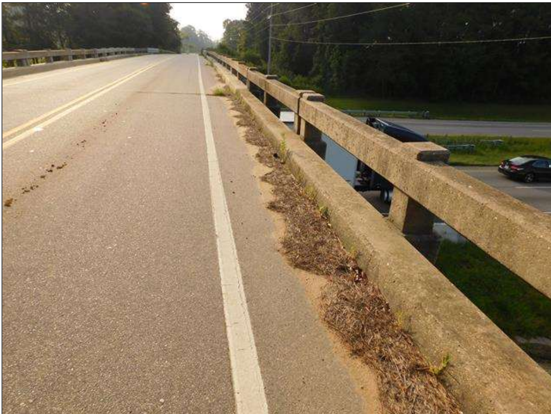
DECK DEBRIS ALONG BOTH CURBS
