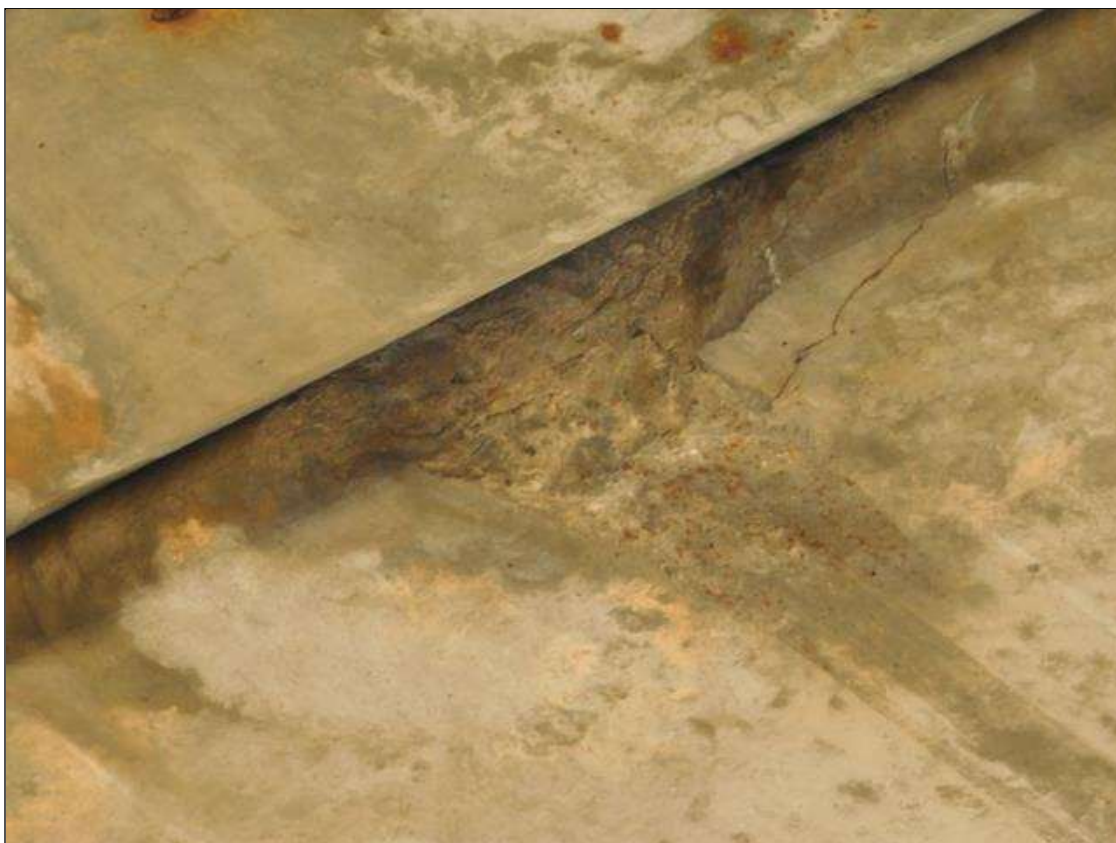
Span 2 Slab 9: LOWER SIDE OF THE SLAB AT THE LEADING CORNER HAS PAST IMPACT DAMAGE, APPROX 4"LINE X UP TO 4"W X UP TO 1"D CENTERED OVER THE RT SOUTHBOUND LANE
