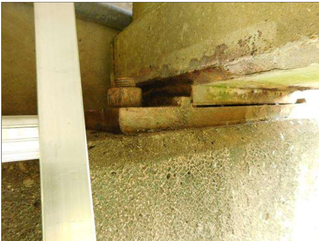
Span 4 Beam 1 Near Bearing: FRECKLED CORROSION
