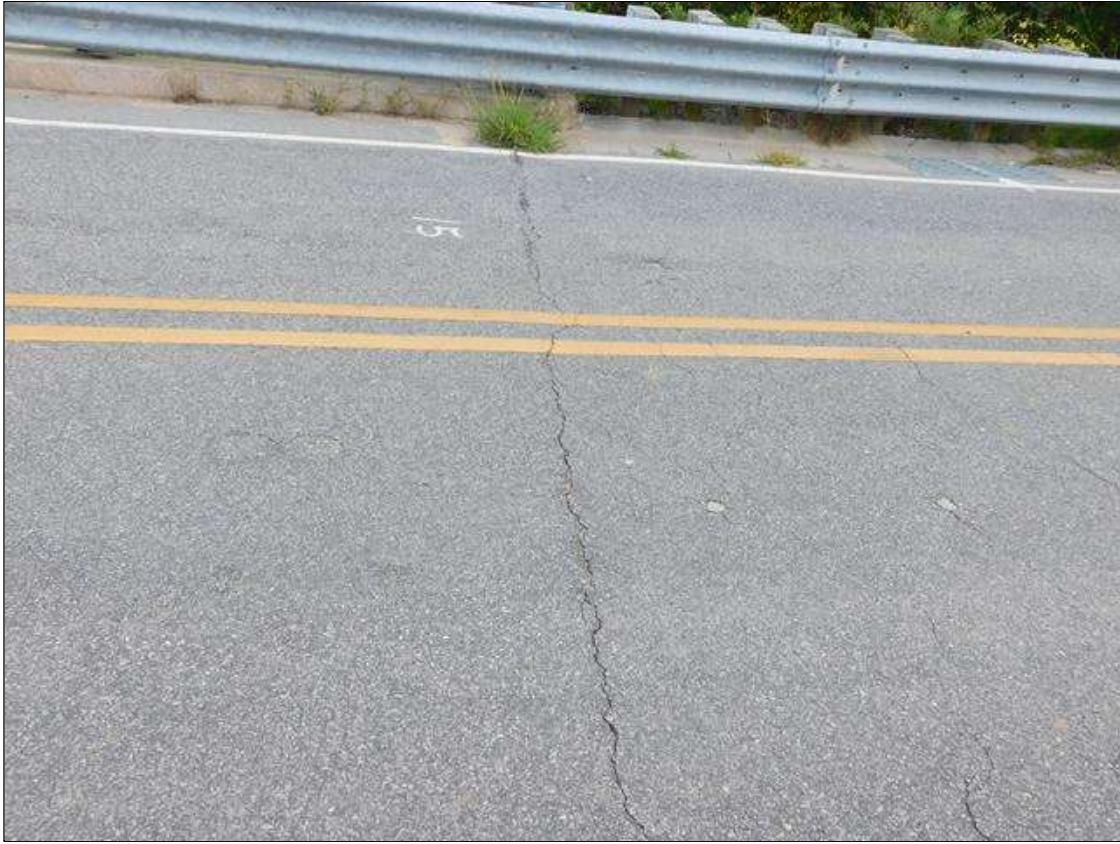
Span 4 Wearing Surface: .005 TO .020 WIDE TRANSVERSE CRACK OVER END BENT 2
