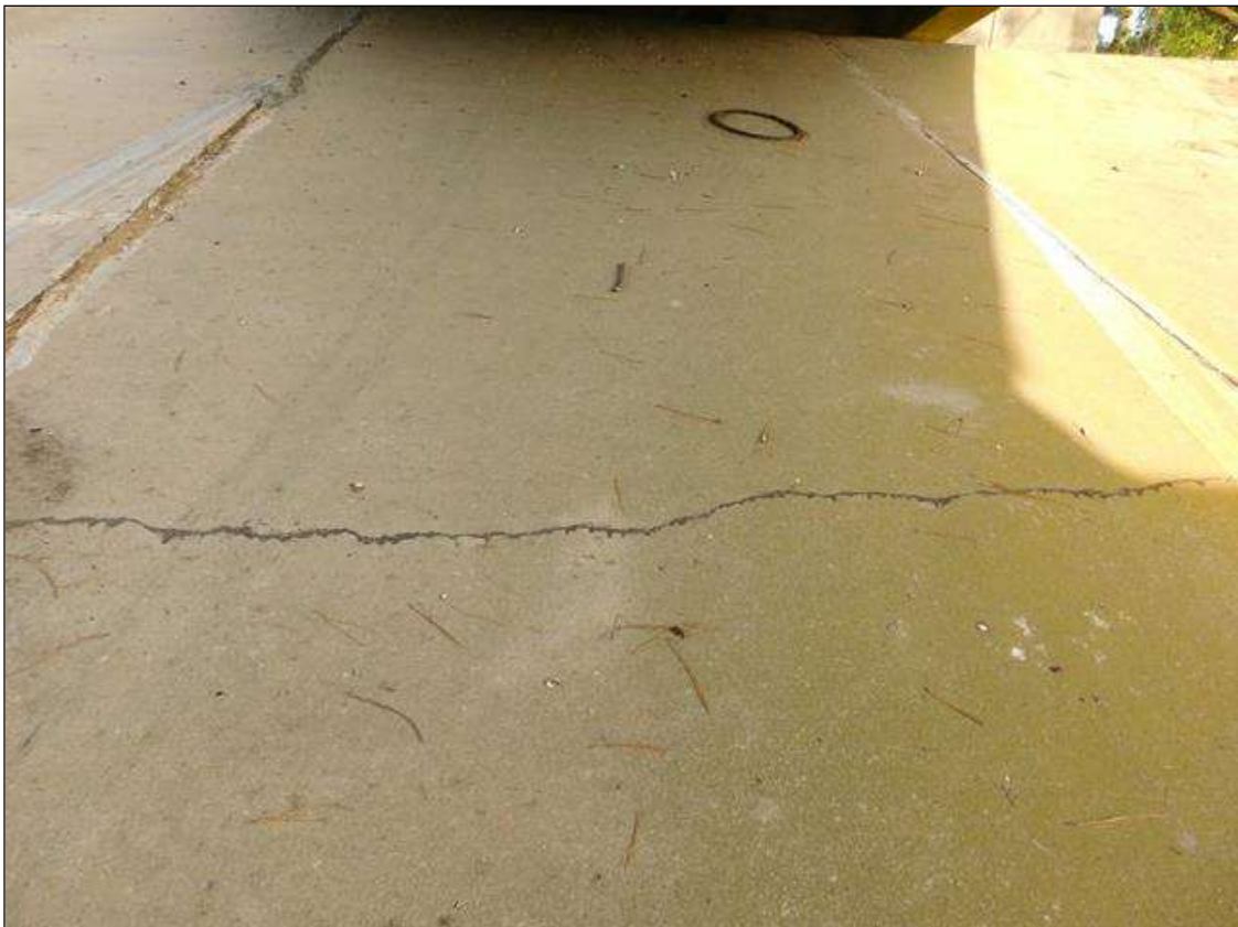
END BENT 1 SLOPE PROTECTION .010 WIDE TRANSVERSE CRACKING 45 FT.
