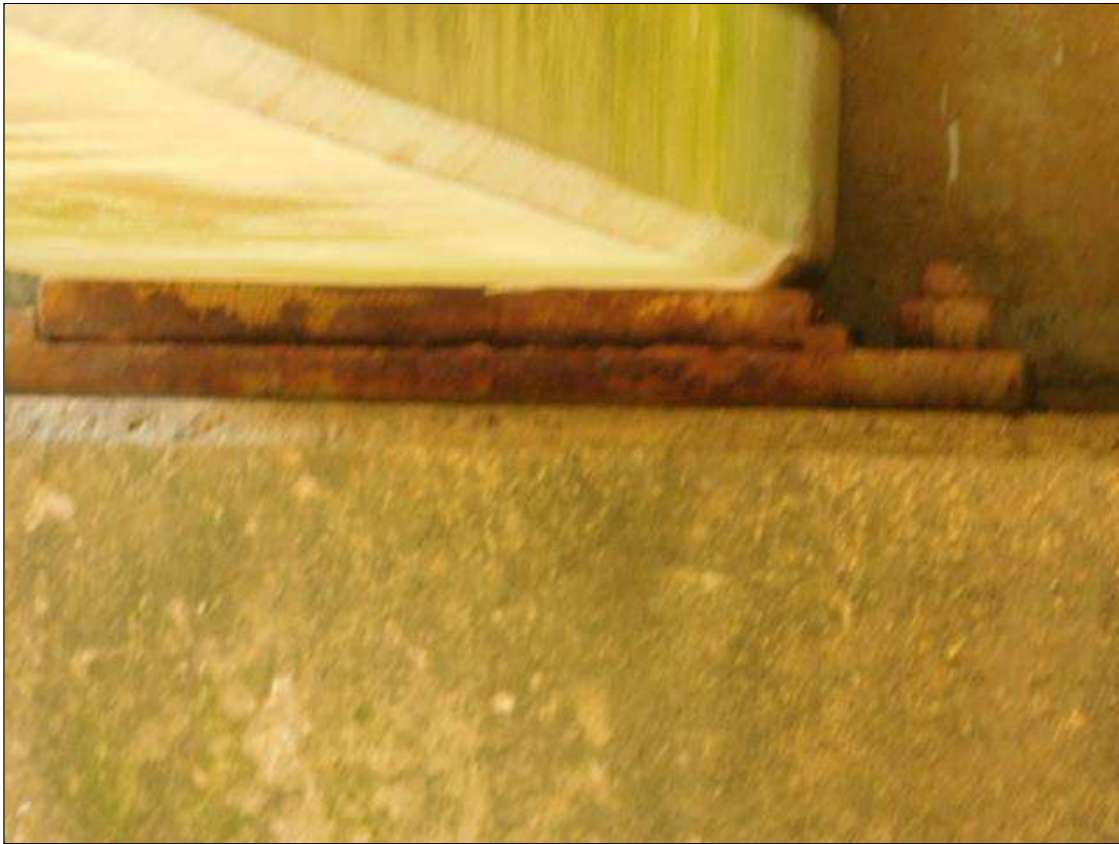
Span 1 Beam 1 Far Bearing: FRECKLED CORROSION
