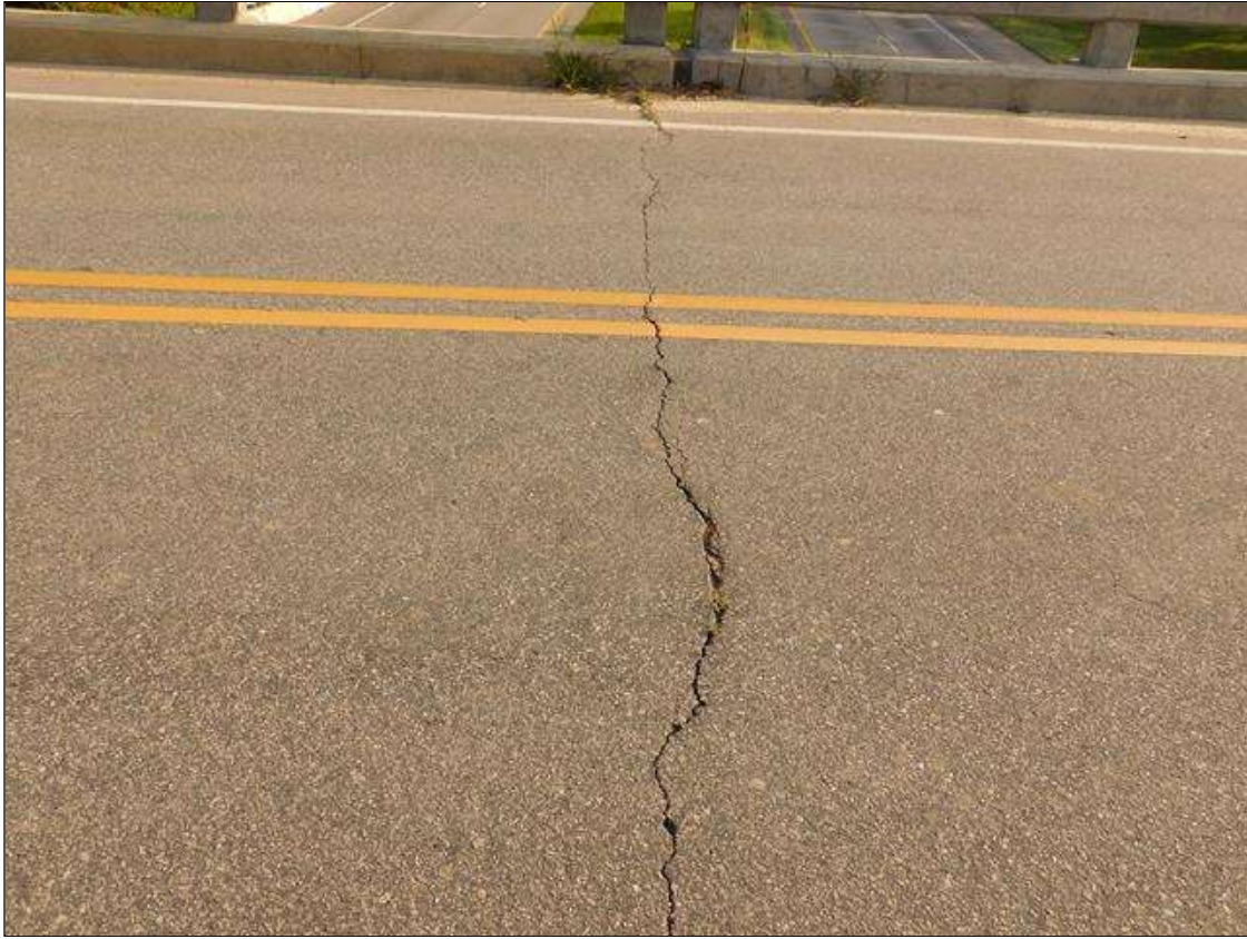
Span 3 Wearing Surface: .005 WIDE TRANSVERSE CRACK OVER BENT 2
