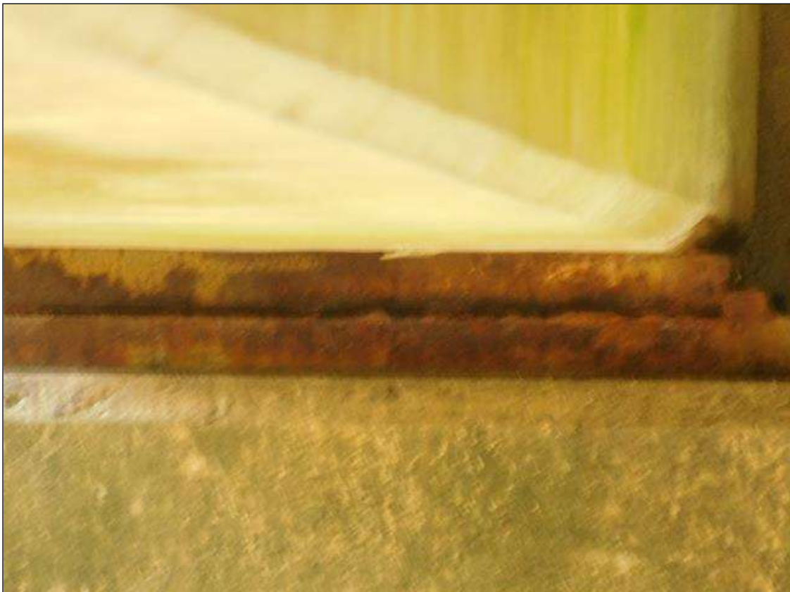
Span 1 Beam 1 Far Bearing: FRECKLED CORROSION
