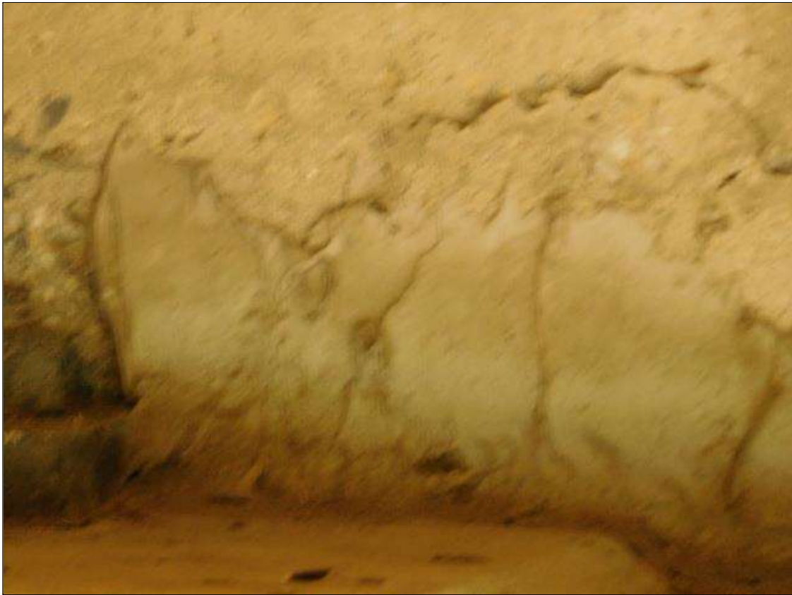
End Bent 1 Abutment/Backwall : BAY 1, SOUND PATCH AT LOWER SIDE AT GIRDER 2
