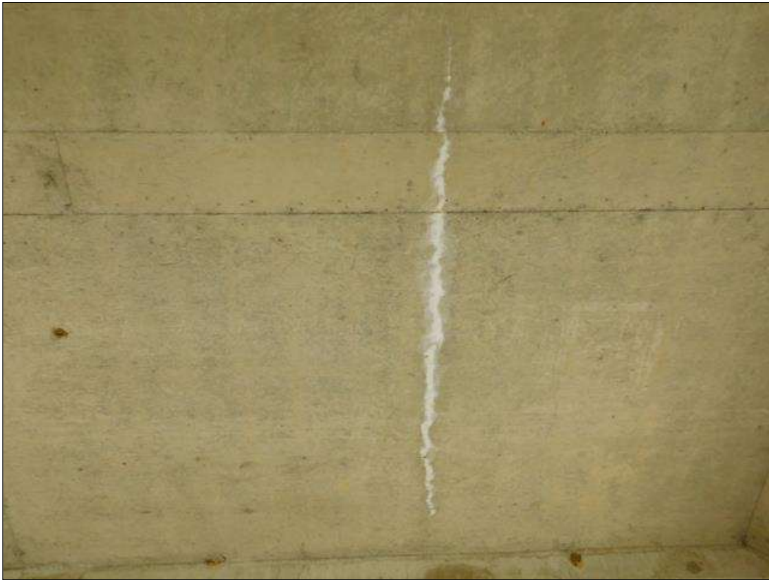
Span 4 Deck: 60 Square Feet of transverse Cracking (RC and Other): Width up to 1/32" with efflorescence near mid-span ON UNDERSIDE OF DECK
