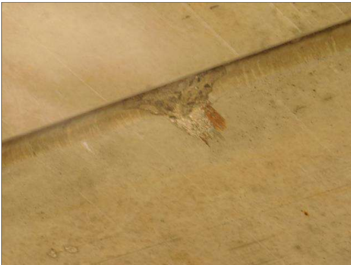
Span 2 Slab 5: LOWER SIDE OF THE SLAB AT THE LEADING CORNER HAS PAST IMPACT DAMAGE, APPROX 2"LINE X UP TO 4"W X UP TO 1"D CENTERED OVER THE RT SOUTHBOUND LANE
