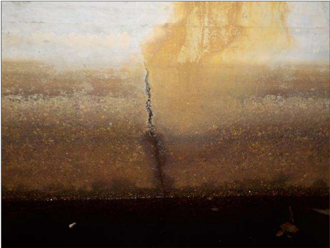
BAREL 3: H/L CRACK W/EFFLO
