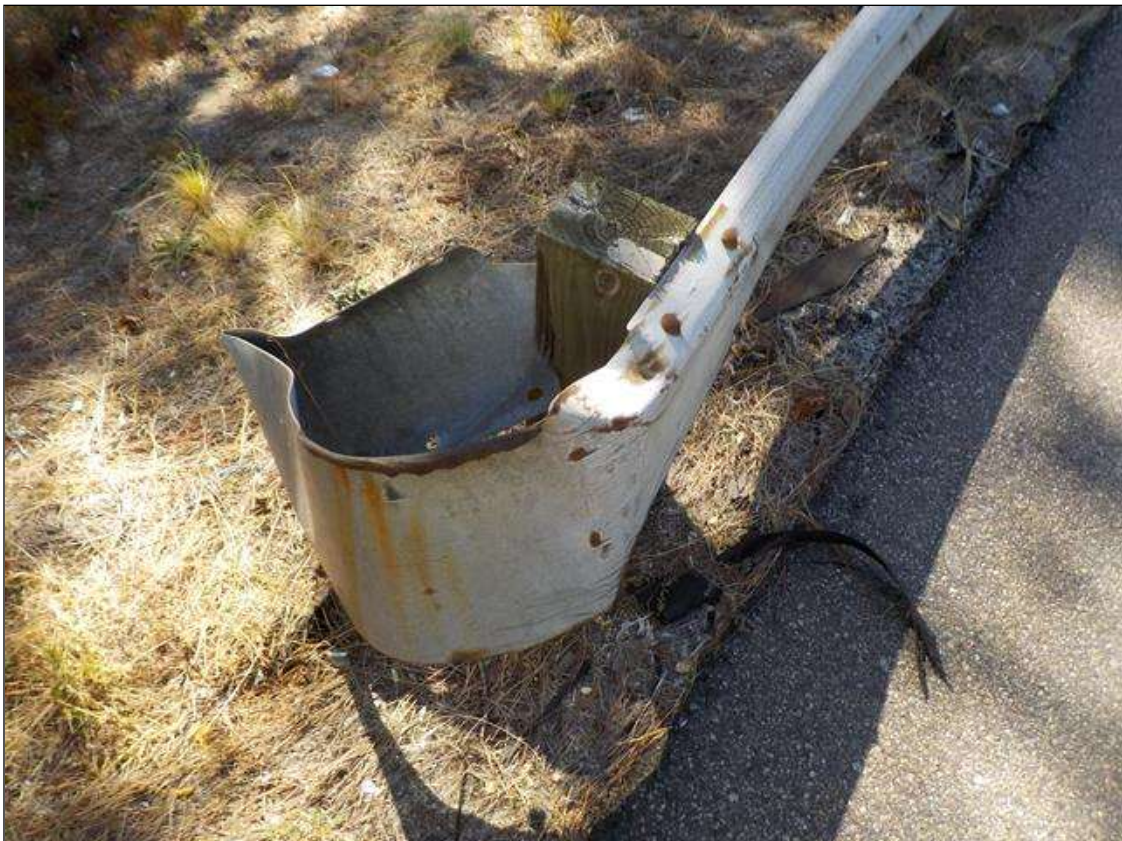
NE GUARDRAIL DAMAGED
