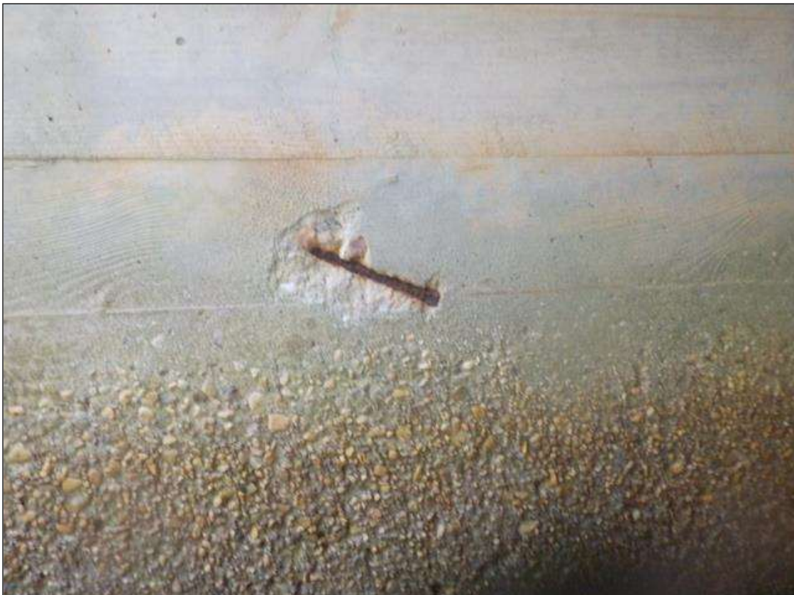
BARREL 1: SPALL NEAR EAST END, W/REBAR
