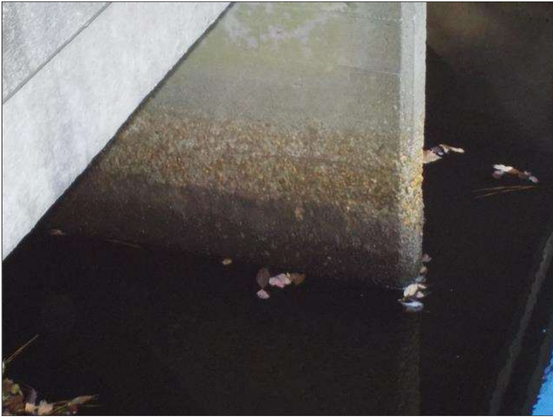
COARSE AGG EXPOSED ON INTERIOR WALL
