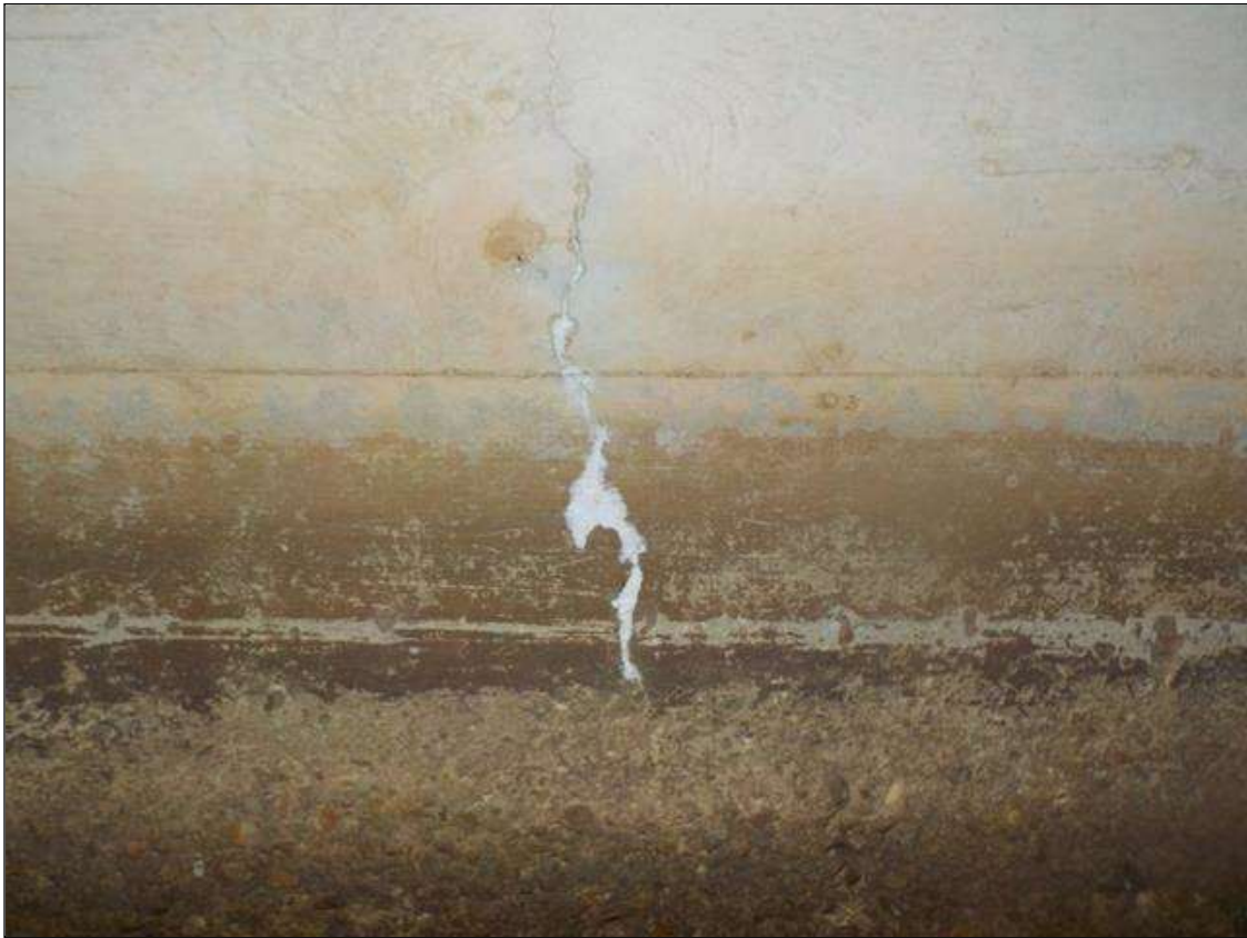
CRACK W/EFFLO, BARREL 1
