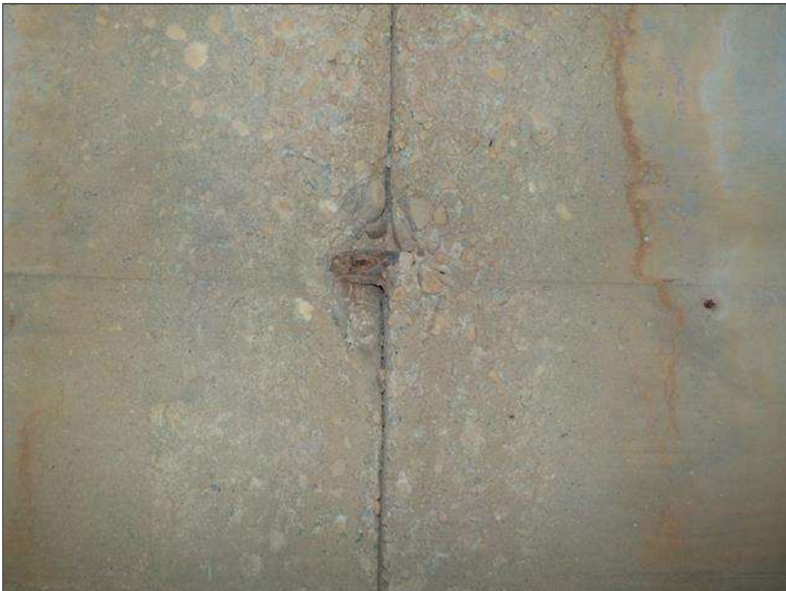
CONSTRUCTION JOINT OPEN TO 1/4" W/EXPOSED REBAR. NO SECTION LOSS IN SPALL, 3"V X 3"W X 1"D
