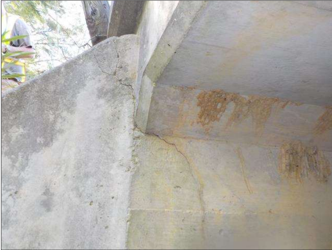
CRACK AT SE WING TO 1/16"
