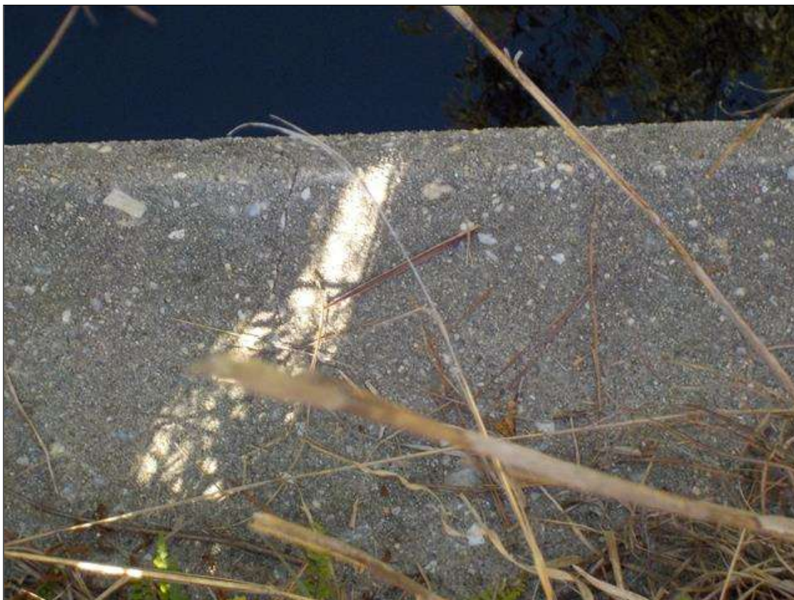
HEADWALL, H/L CRACK
