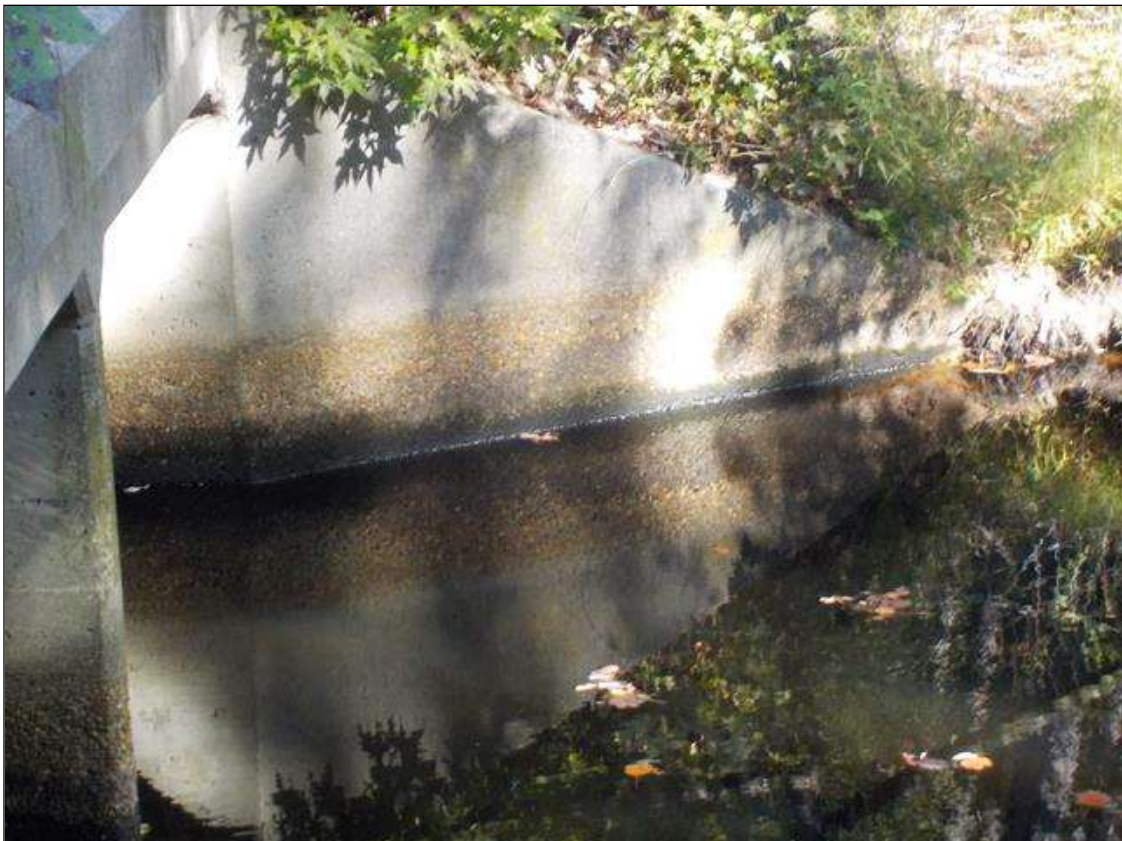
COARSE AGG EXPOSED ON WINGWALL
