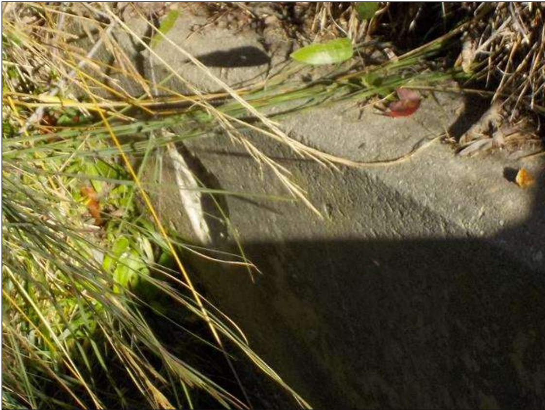
SPALL, NW WINGWALL, 6"DIA. X 1"D
