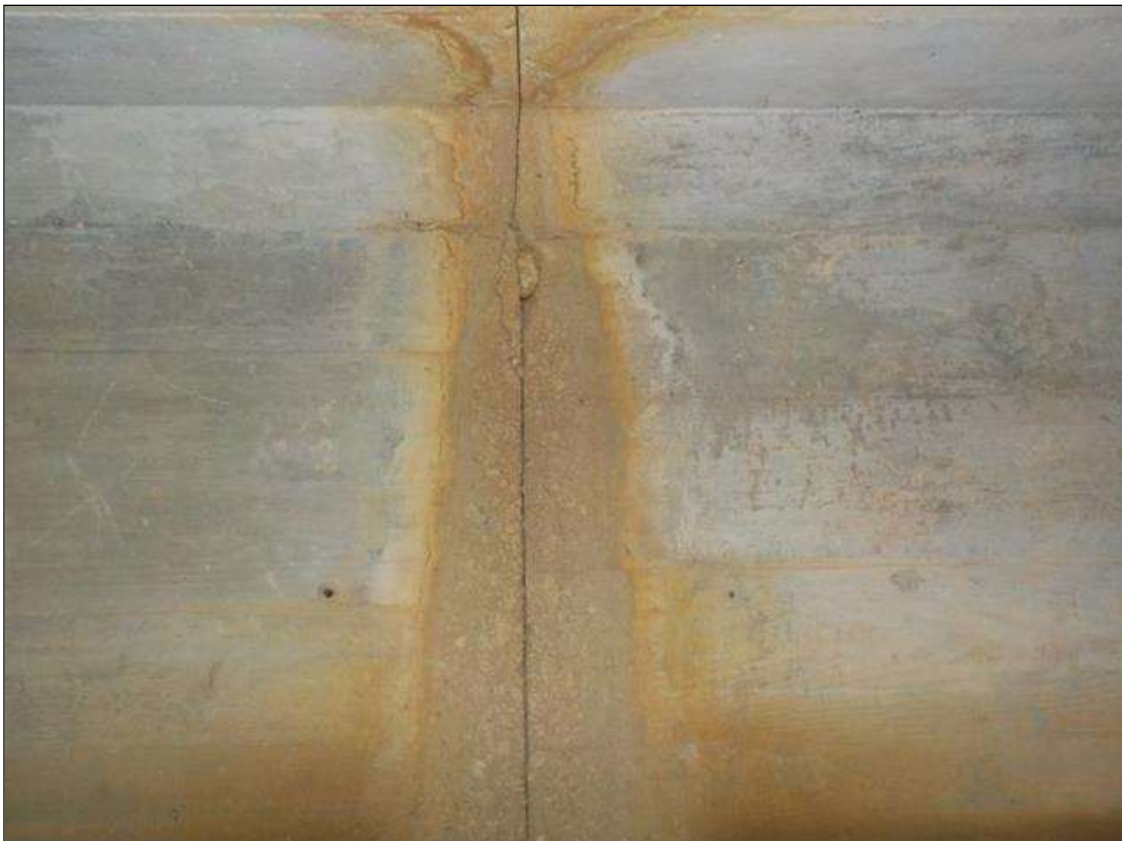
BARREL 1: CONSTRUCTION JOINT W/RUST
