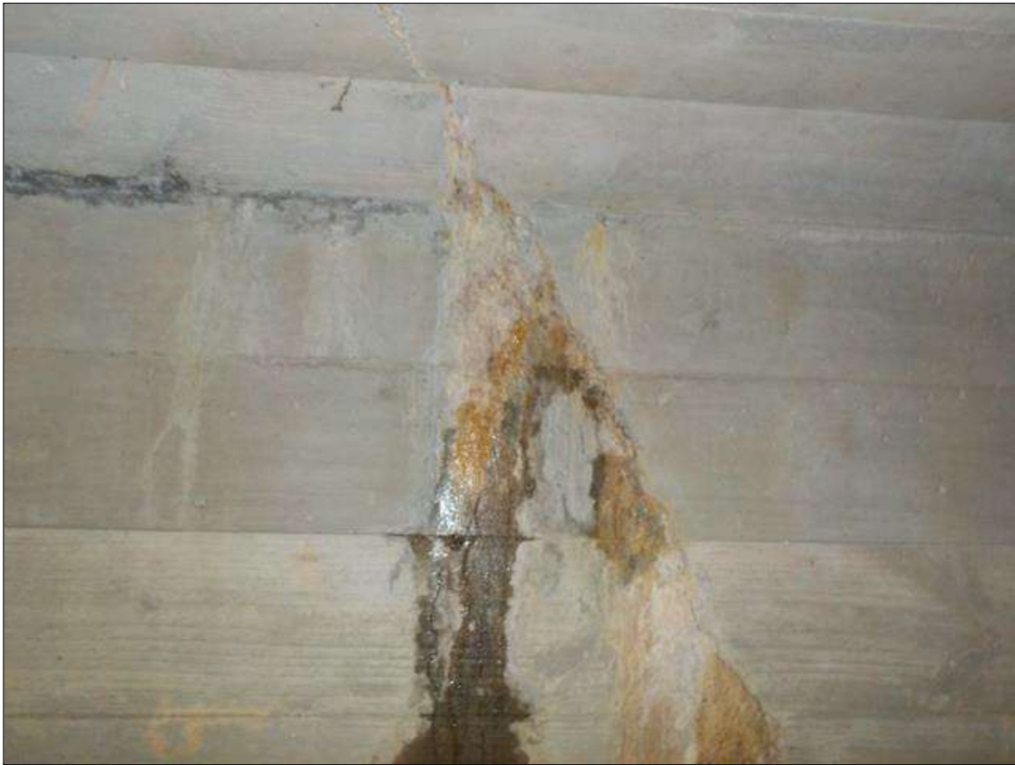
BARREL 2: CRACK W/EFFLO
