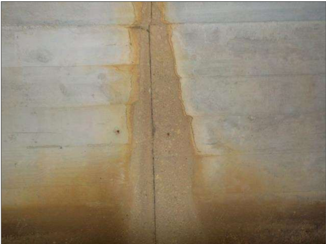
BARREL 3: CONSTRUCTION JOINT OPEN TO 1/4"
