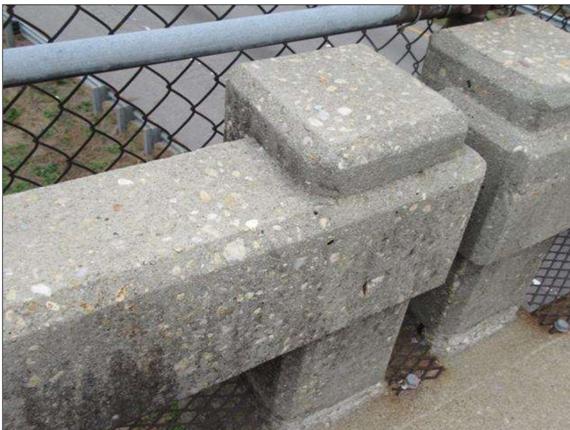
SPAN 1 LEFT RAIL HAS EXPOSED AGGREGATE
