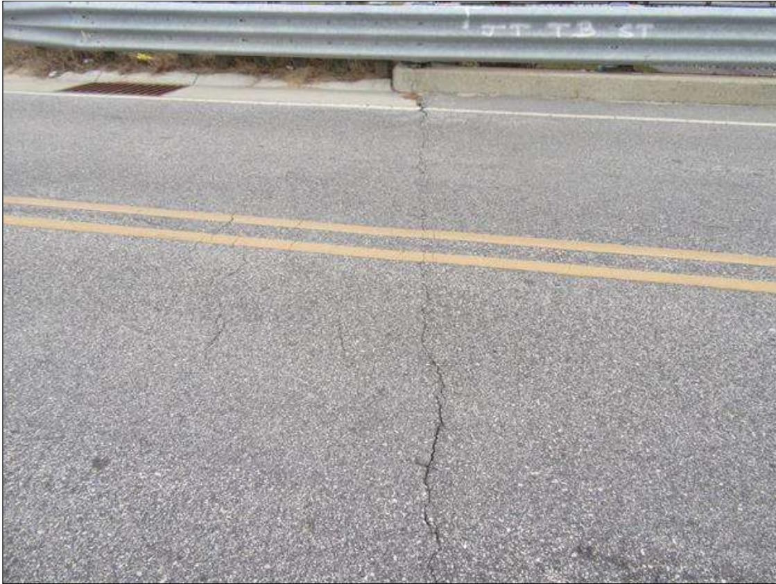
Span 1 Wearing Surface: 1/8" WIDE TRANSVERSE CRACK OVER END BENT 1
