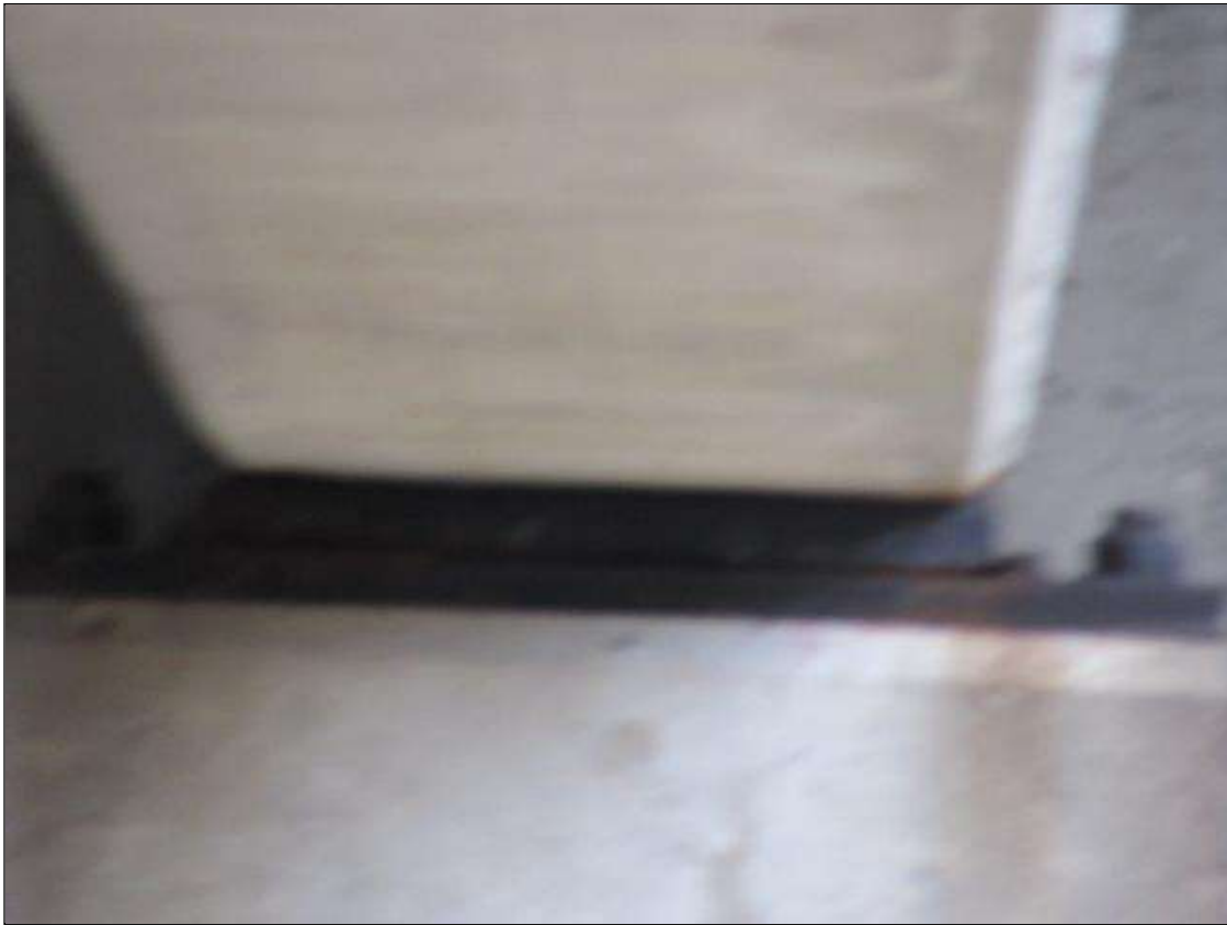
SPAN 1 BEAM 4 FAR BEARING CLEANED AND PAINTED WITH BLACK MAX, ALL BEARINGS IN SPANS 1 AND 4 SIMILAR
