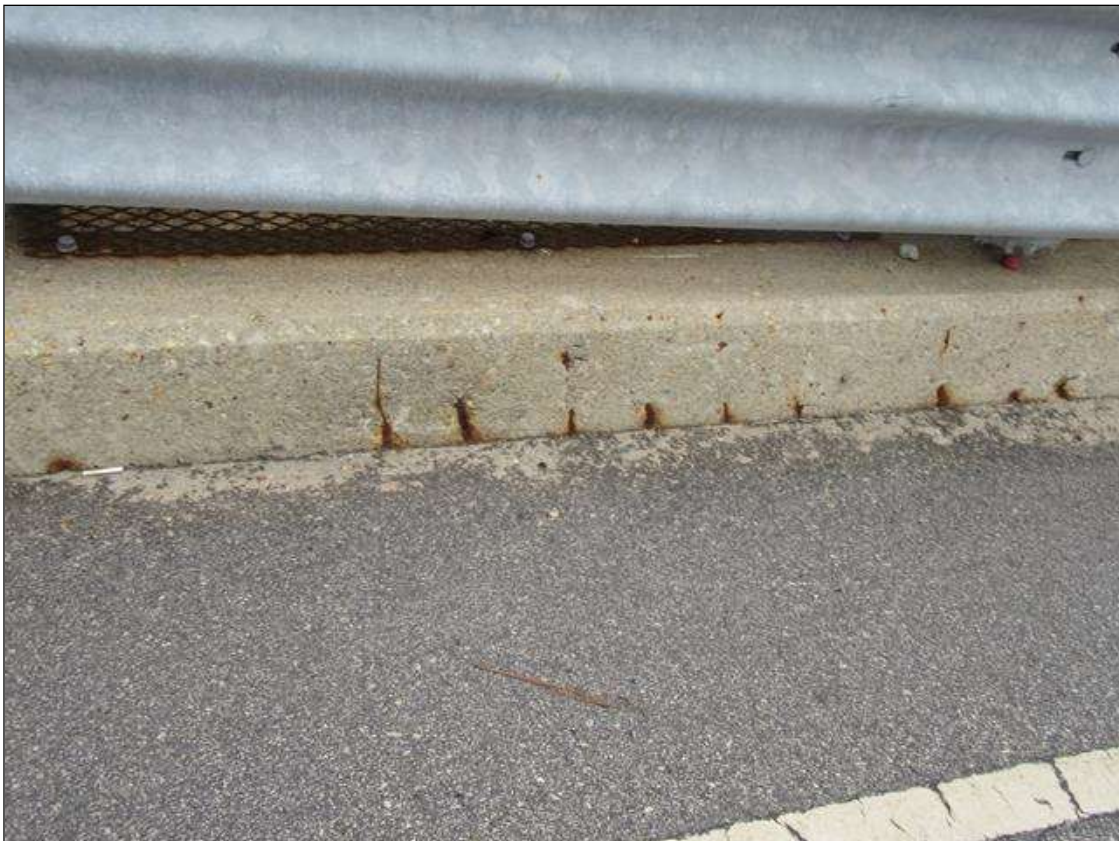
Span 1 Right Bridge Rail: SURFACE SPALLS 18 WITH EXPOSED REBAR IN RIGHT CURB
