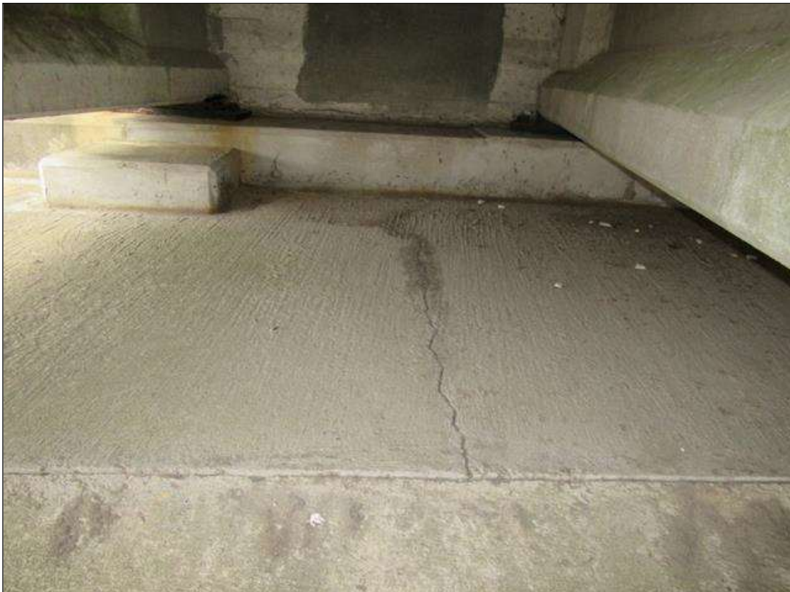
END BENT 1 TOP OF SLOPE AT BAY 1 6 FT. LONG X 1/4" WIDE LONGITUDINAL CRACK
