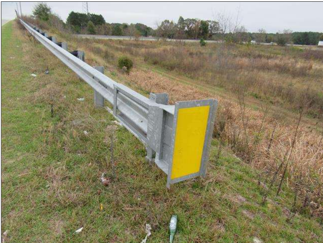
GUARDRAIL END TERMINAL
