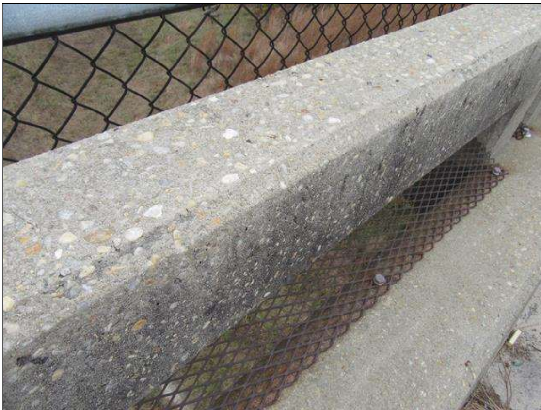
SPAN 4 LEFT RAIL HAS EXPOSED AGGREGATE
