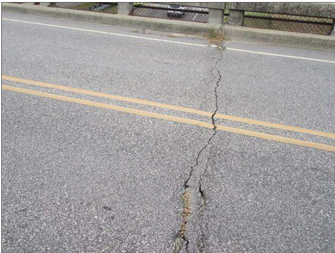
Span 1 Wearing Surface: 1/4" WIDE TRANSVERSE CRACK OVER BENT 1
