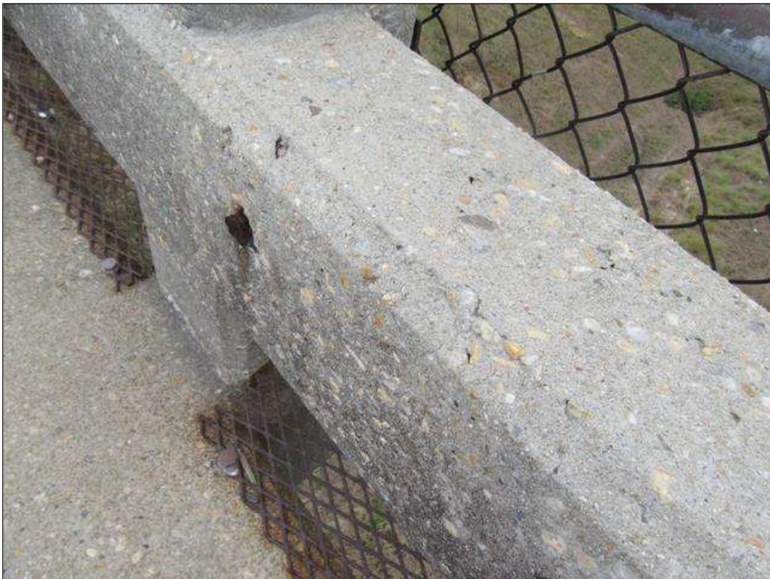
SPAN 4 RIGHT RAIL HAS EXPOSED AGGREGATE
