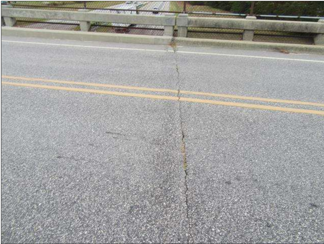
Span 3 Wearing Surface: 3/16" WIDE TRANSVERSE CRACK OVER BENT 3
