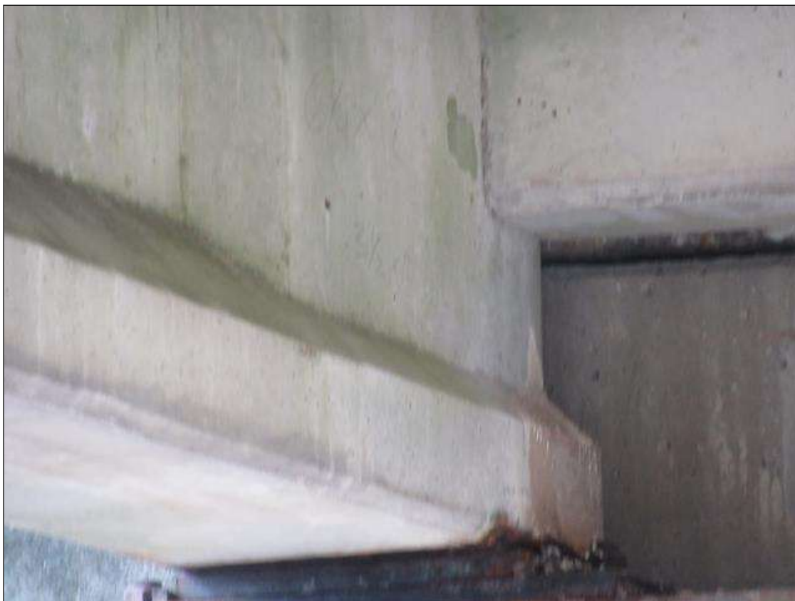
Span 1 Beam 1: SOUND PATCH FAR END ON BAY1 SIDE AT BENT 1
