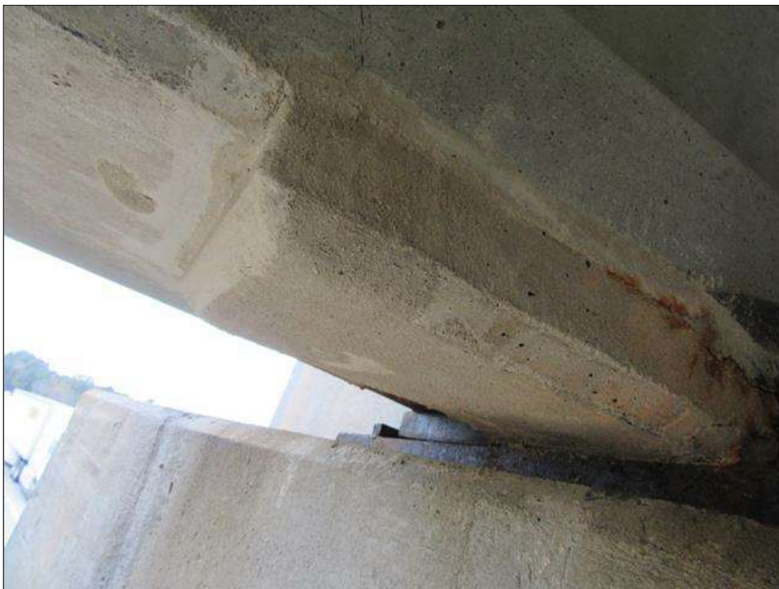
Span 4 Beam 4: SOUND PATCH IN BOTTOM FLANGE NEAR END AT BENT 3, PRIORITY MAINTENANCE REPAIR.
