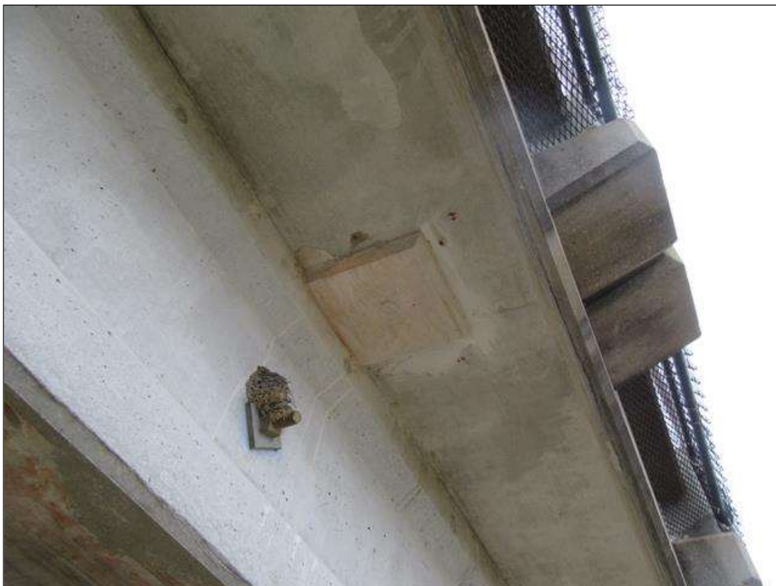
Span 1 Deck: RIGHT DECK OVERHANG SOUND PATCH AT MID SPAN
