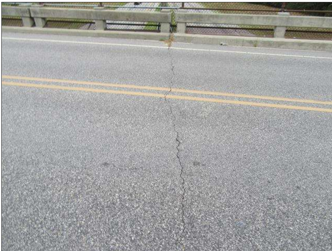
Span 2 Wearing Surface: 1/8" WIDE TRANSVERSE CRACK OVER BENT 2
