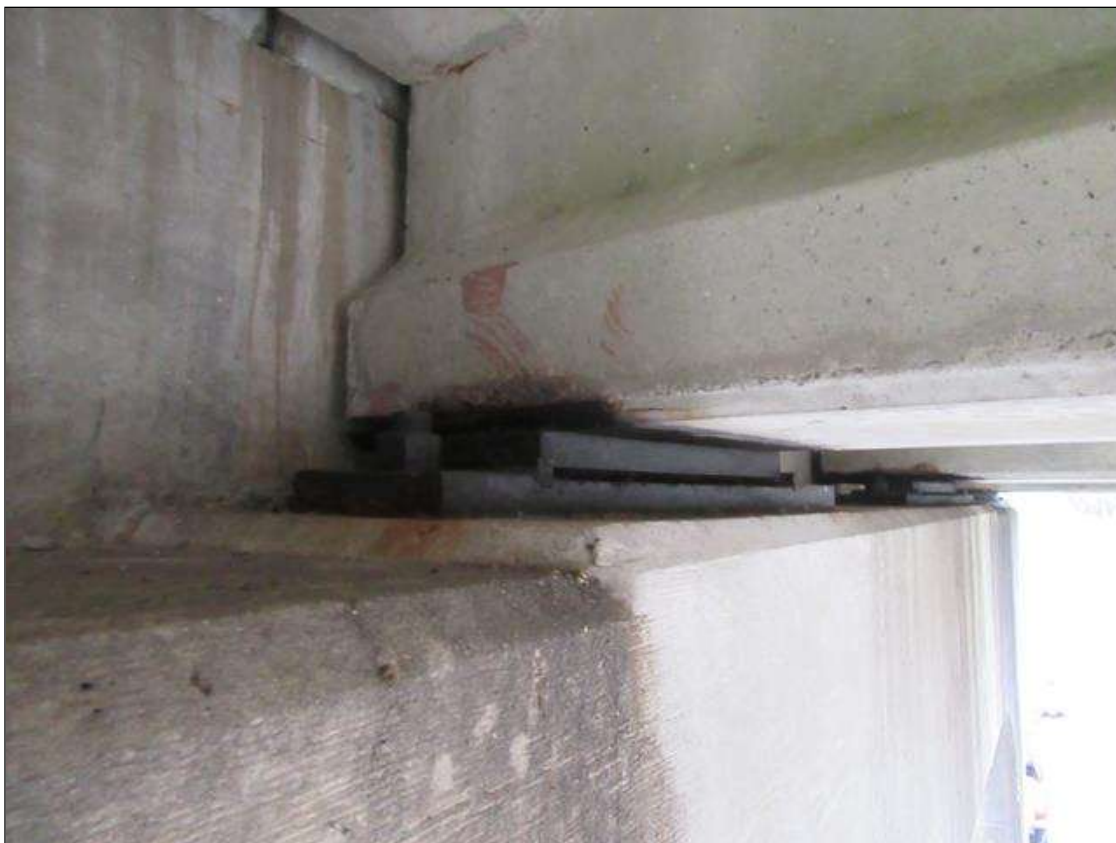
SPAN 4 BEAM 4 NEAR BEARING CLEANED AND COATED WITH BLACK MAX, ALL BEARINGS IN SPANS 1 AND 4 ARE SIMILAR
