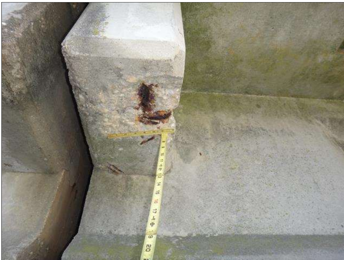
Span 4 Deck: diaphragm at right overhang over bent 3, spall/delamination [10in x 10in x 3in deep] with one [1] exposed longitudinal rebar and one [1] exposed vertical stirrup [section loss up to 1/16in]
