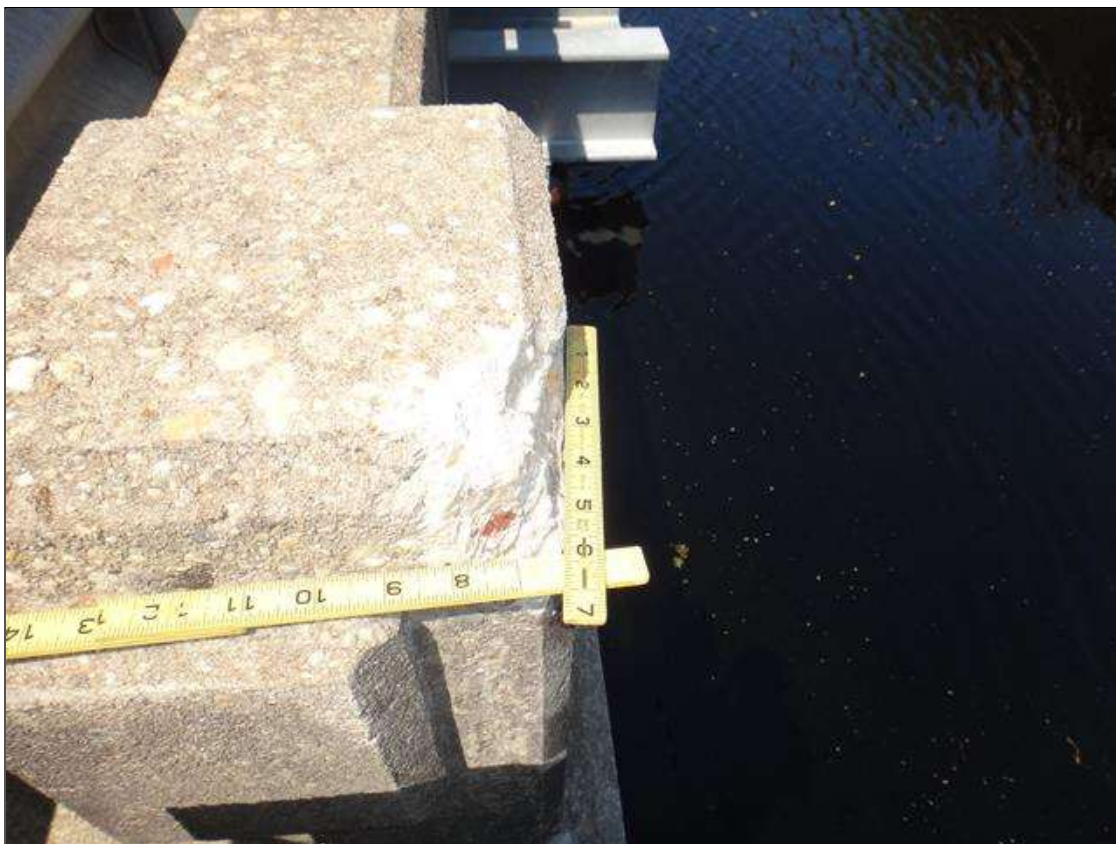
Span 3 Right Bridge Rail: at rail post 4, spall [7in x 5in x 1in deep] [similar at rail post 6]
