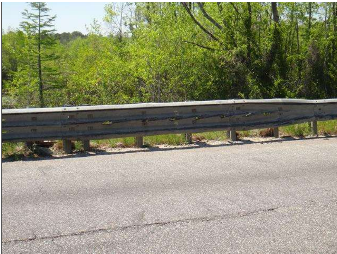
Northwest guardrail: at North approach, vehicular impact damage [25ft long] with multiple gouges [up to 5in x 3in]
