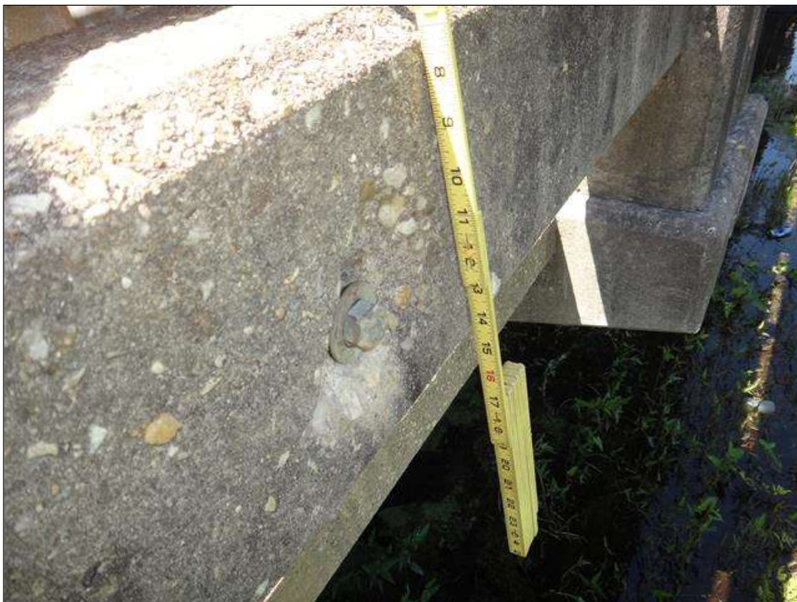
Span 1 Right Bridge Rail: along length of rail at guardrail connections, multiple spalls [up to 5in diameter x up to 1in deep]
