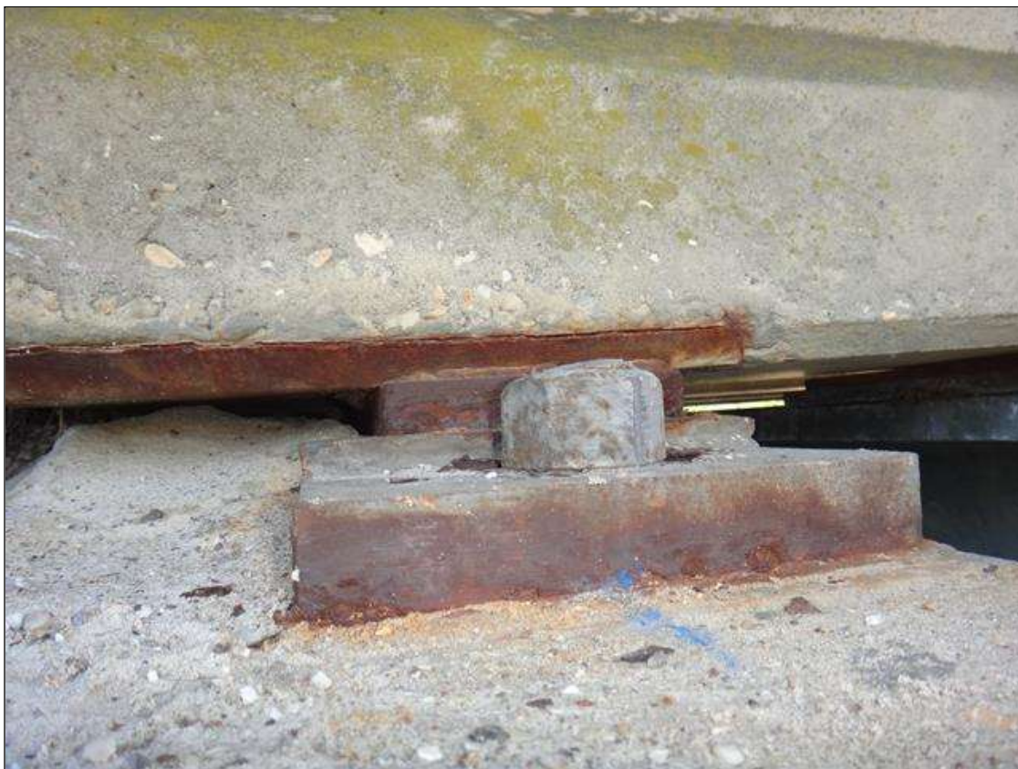
Span 4 Beam 4 Near Bearing: active surface corrosion [no section loss noted]
