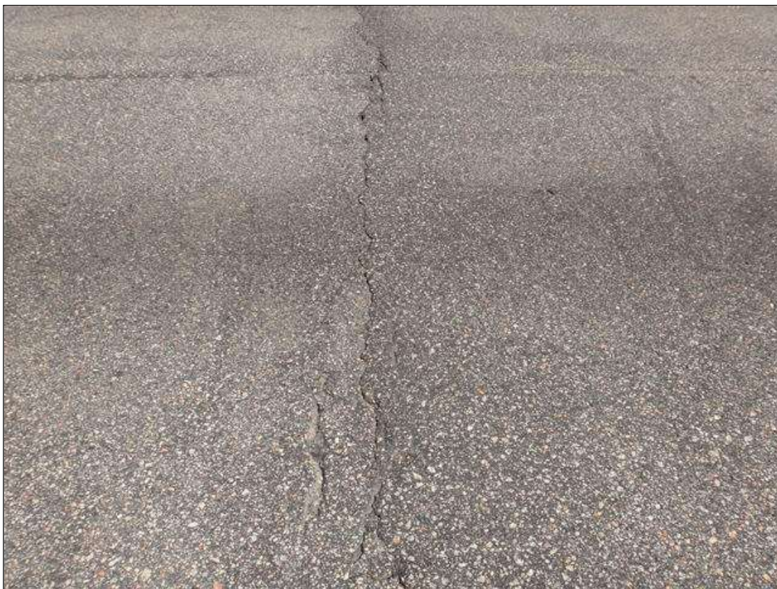
Span 4 Wearing Surface: asphalt over end bent 2, multiple transverse cracks [up to full width x up to 1/2in] with edge spalling [up to 1in]
