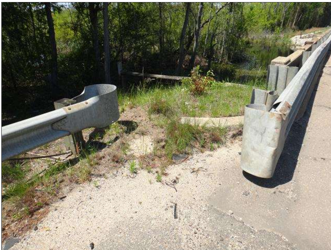
Southwest corner [guardrail not attached to bridge rail]
