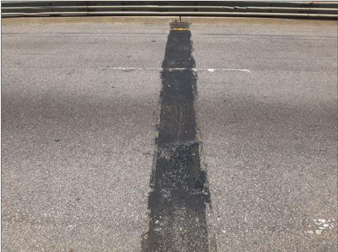
asphalt over bent 2
