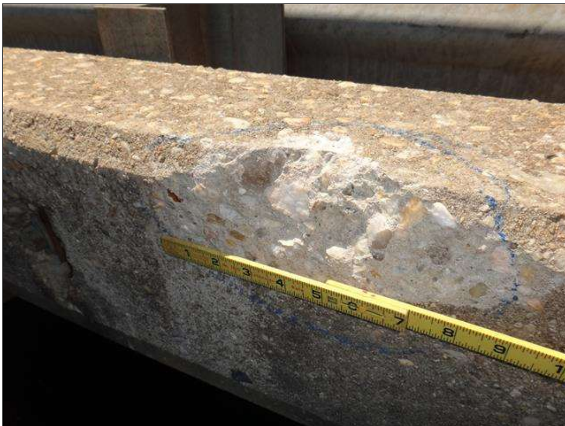
Span 3 Right Bridge Rail: at far third, spall [8in x 4in x 1in deep]
