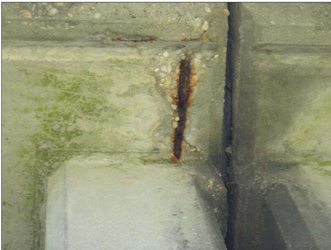
Span 3 Deck: at right overhang over bent 3, spall [10in x 4in x up to 1-1/2in deep] with one [1] exposed rusted reinforcing [section loss up to 1/16in]
