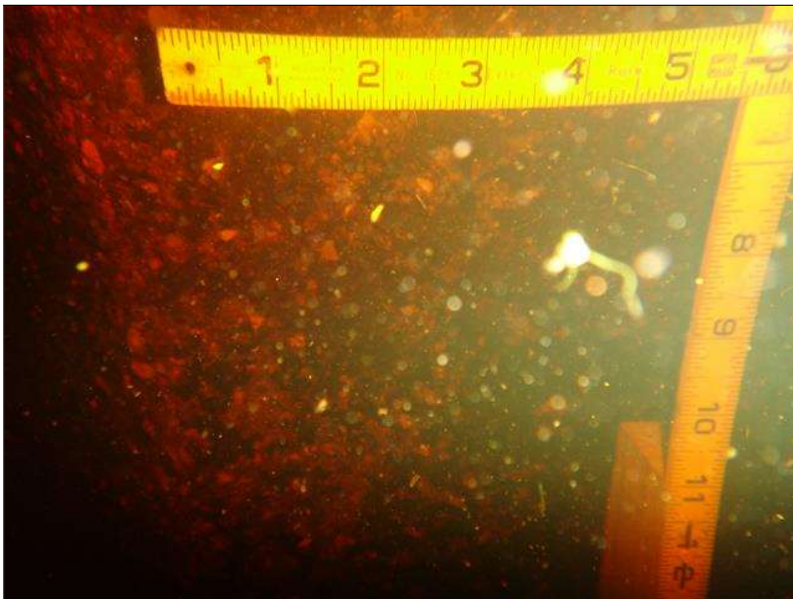
Bent 2 Pile 2: at waterline down 18in, minor abrasion [up to 1/16in deep]
