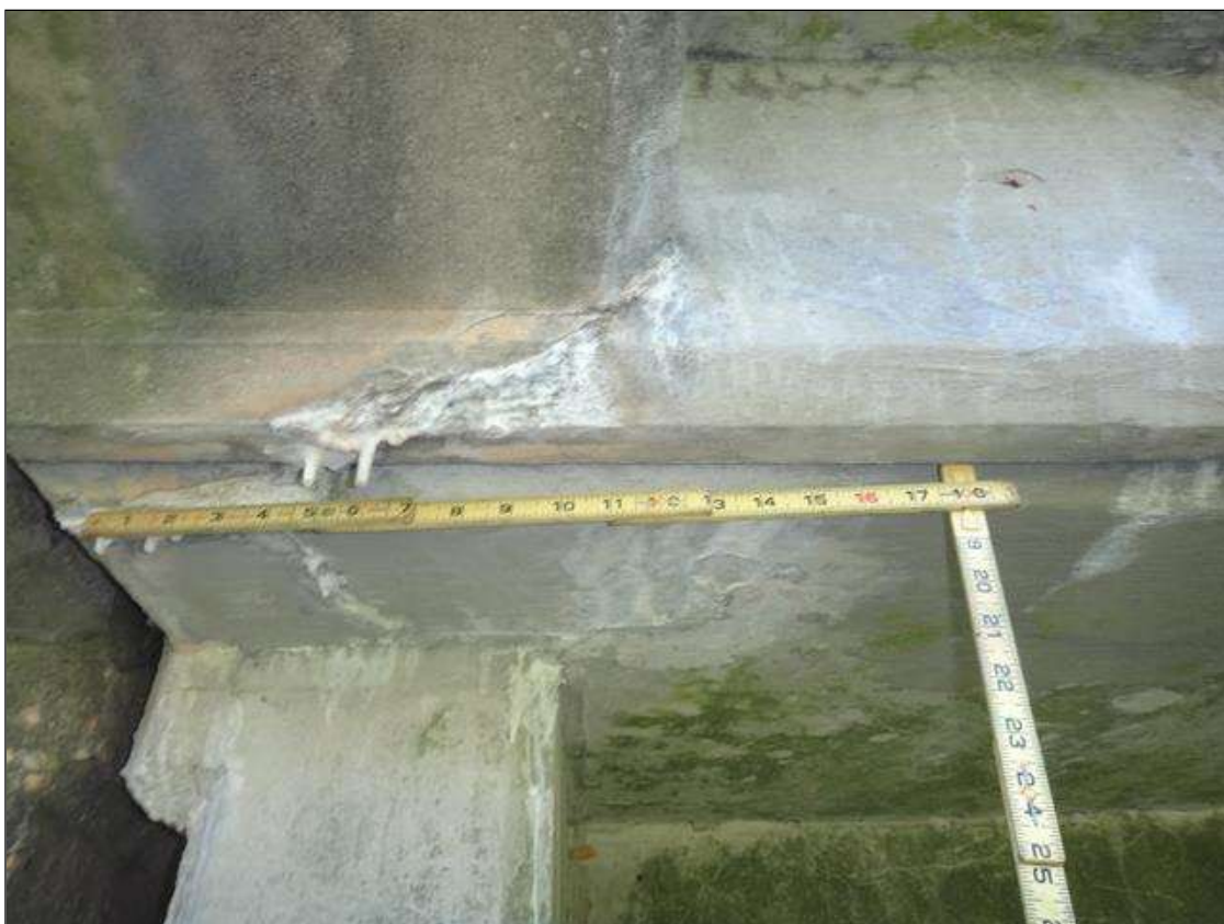
Span 1 Deck: left overhang at bent 1, efflorescence buildup
