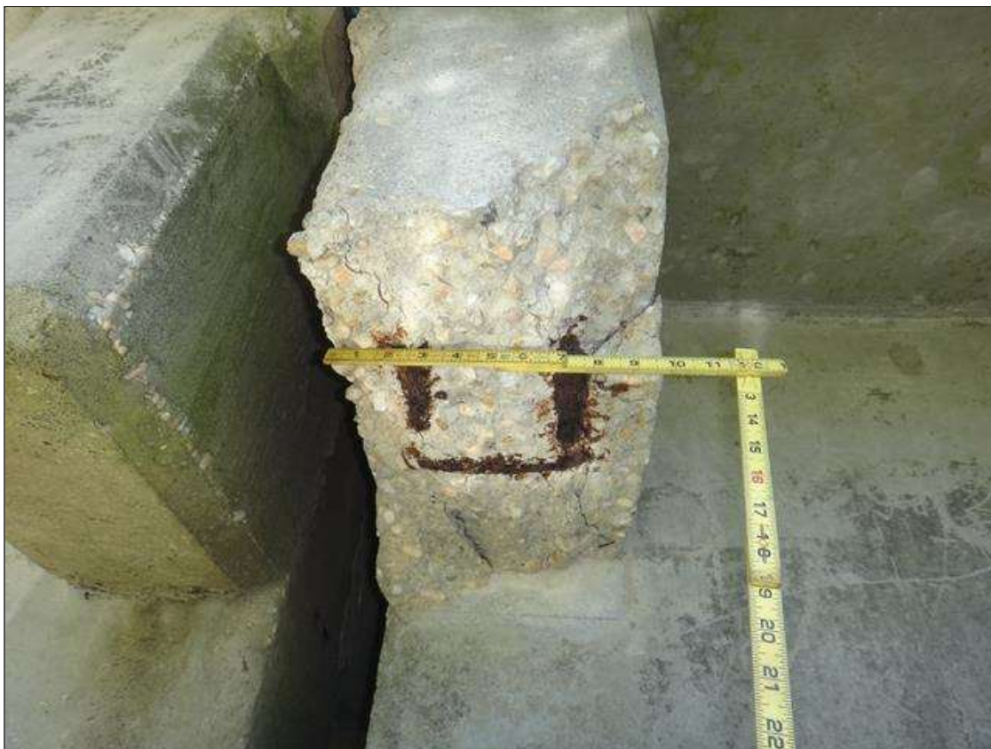
Span 2 Deck: at right overhange over bent 1, spall/delamination [20in x 10in x up to 3in deep] with three [3] exposed rusted reinforcing [section loss < 1/16in]
