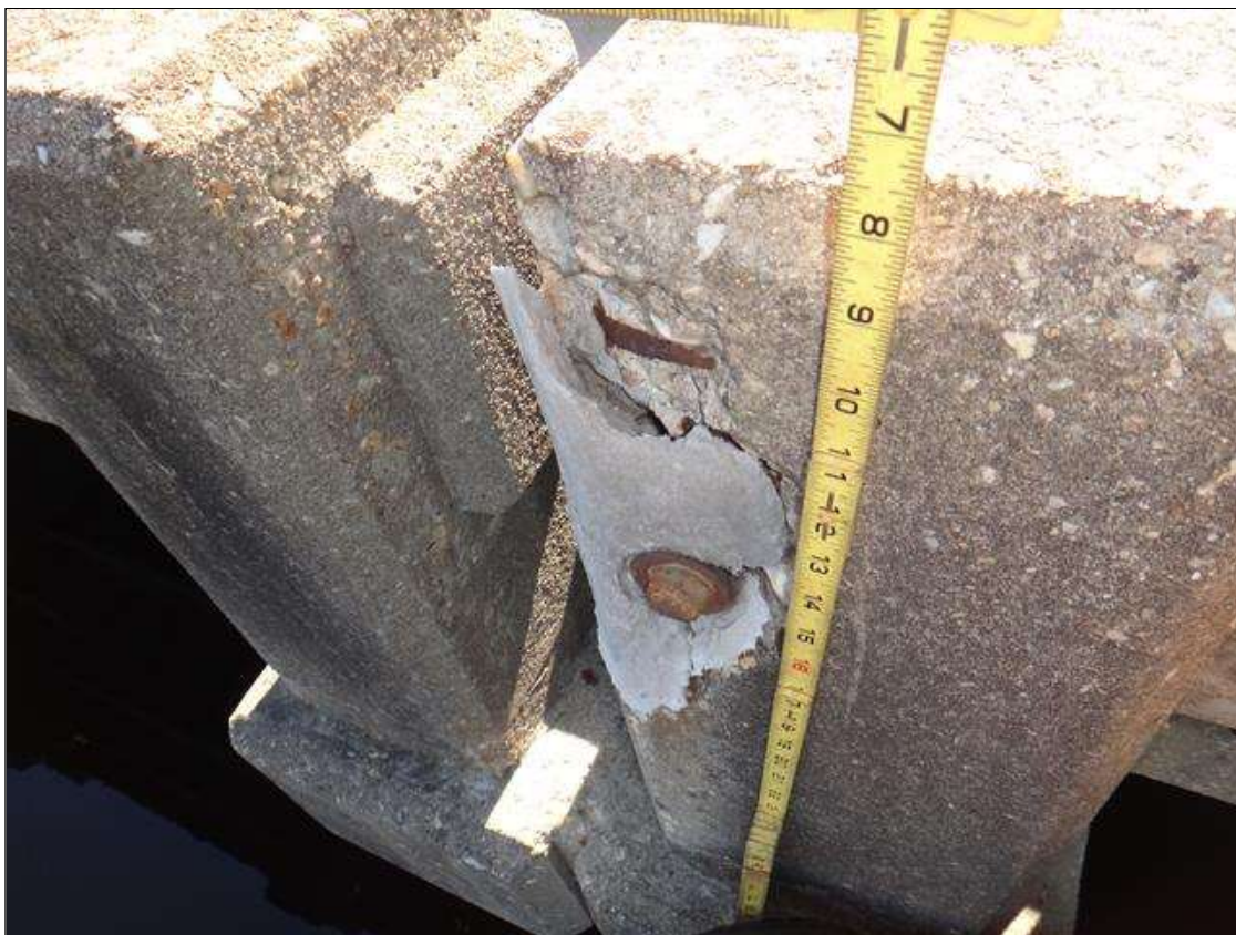
Span 3 Left Bridge Rail: West face at rail post 3, unsound patch [14in x 5in]
