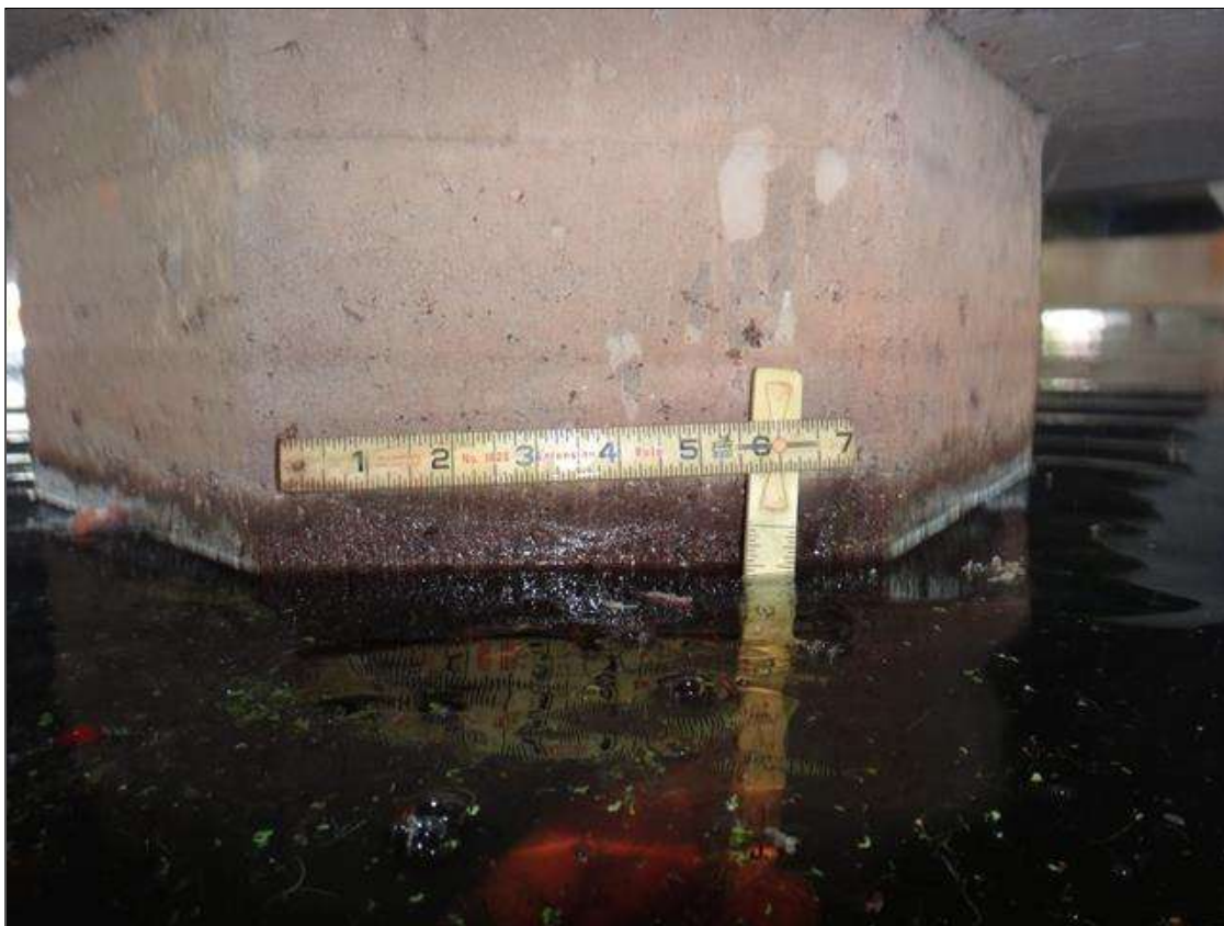
Bent 3 Pile 2: at waterline down 18in, minor abrasion [up to 1/16in deep]
