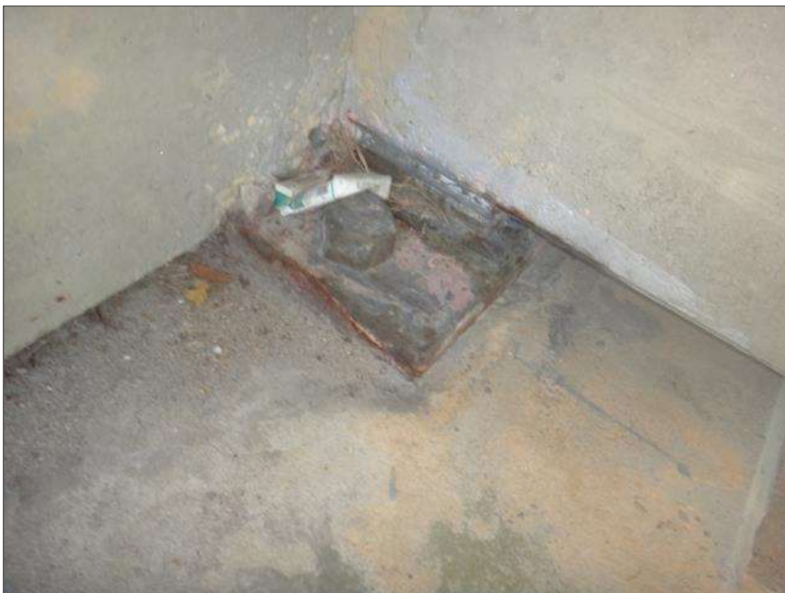
Span 4 Beam 1 Far Bearing: active surface corrosion [no section loss noted]
