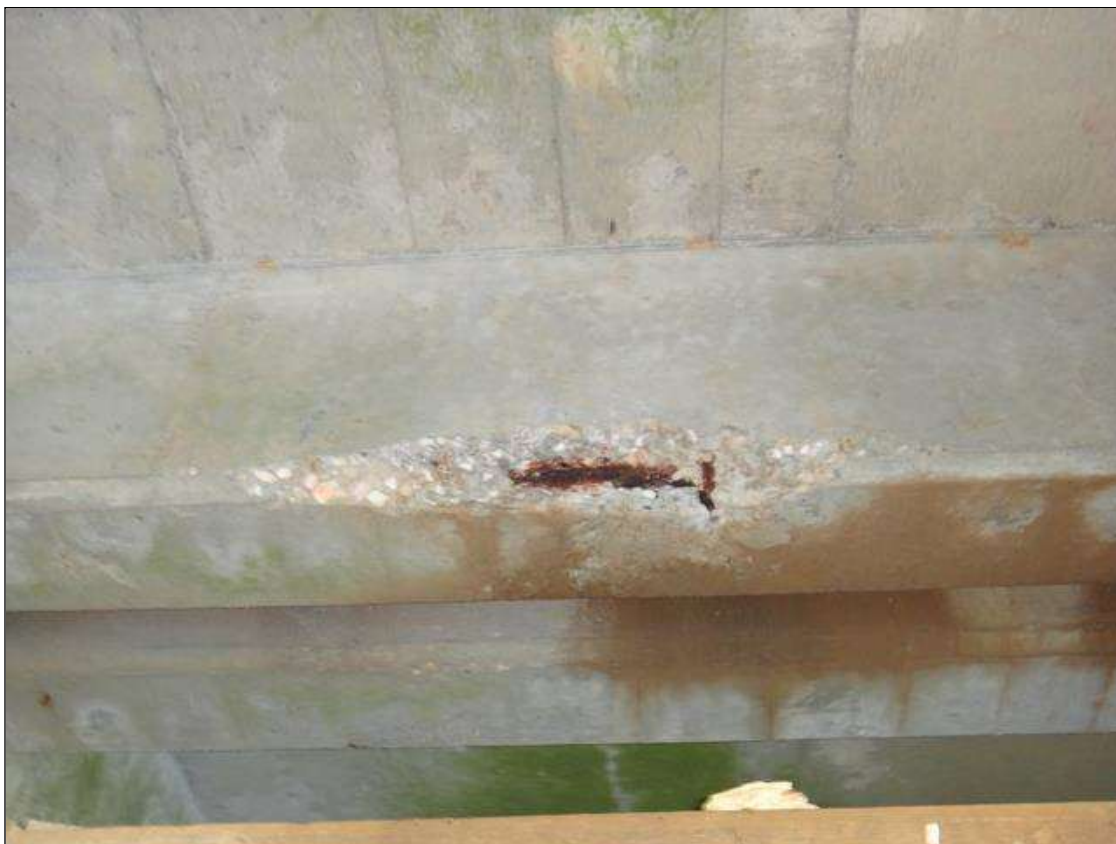
Span 3 Beam 1: North face at lower edge of diaphragm between beams 1 and 2 at near end, spall [24in x 6in x up to 3in deep] with one [1] exposed rusted reinforcing [section loss up to 1/16in]
