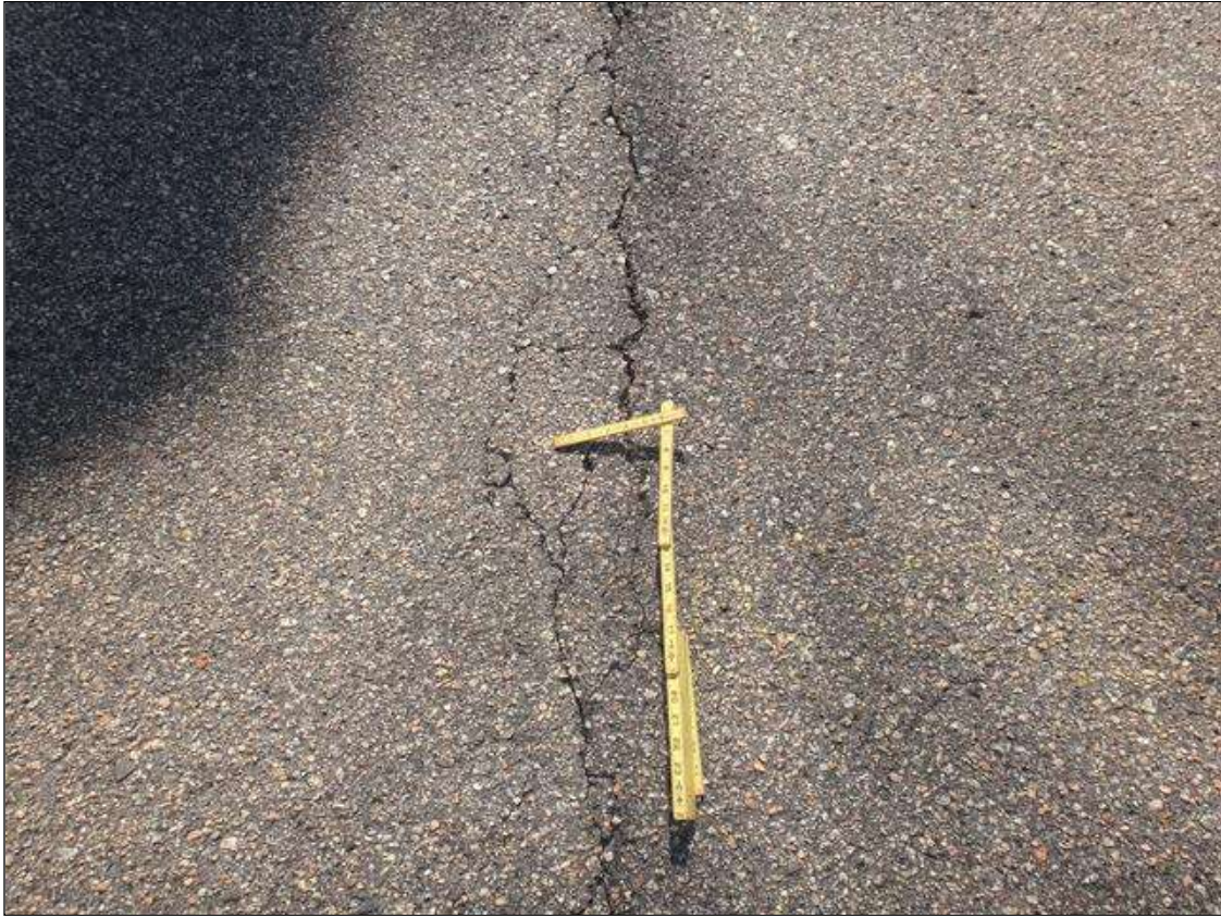
Span 4 Wearing Surface: asphalt over End Bent 2, multiple transverse cracks [up to full width x up to 1/4in] with edge spalling [up to 1in]
