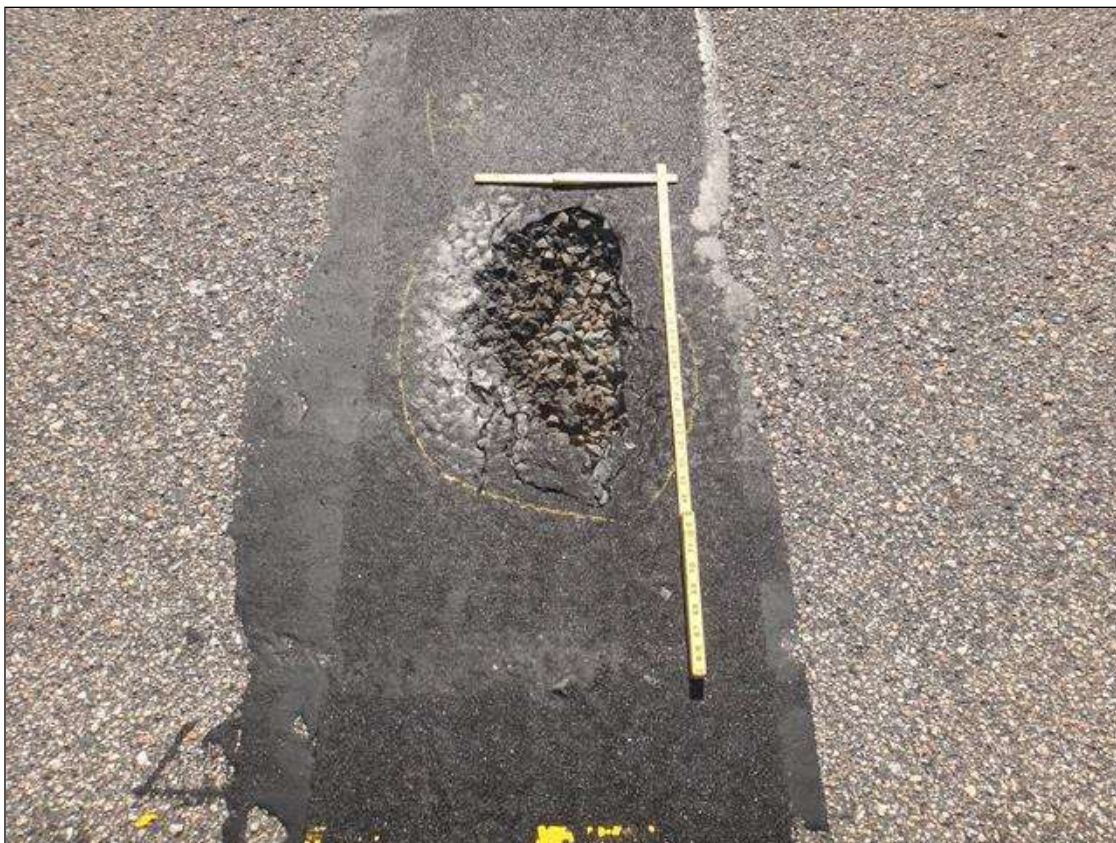
Span 2 Wearing Surface: asphalt over bent 2, one [1] pothole in left travel lane and one [1] pothole in right travel lane [18in x up to 12in x up to 2-1/2in deep]
