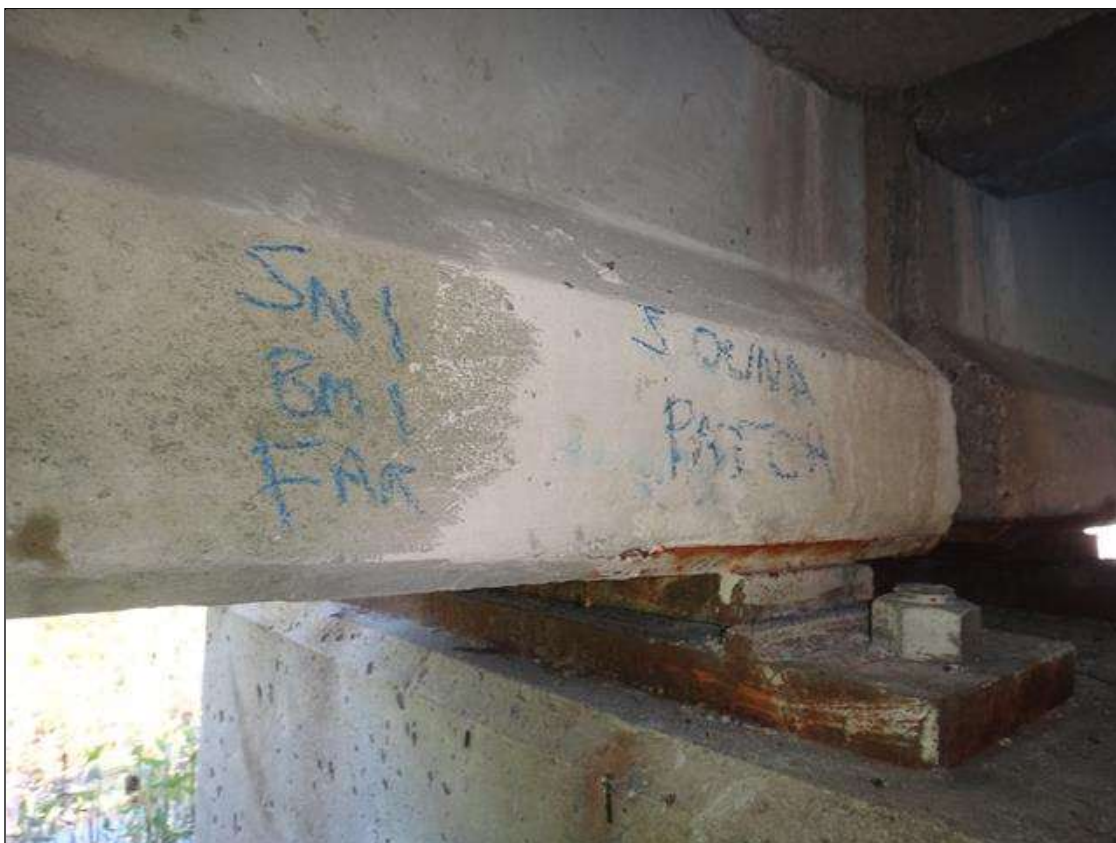
Span 1 Beam 1: at far end 1ft from bent 1, sound patch [4in diameter]
