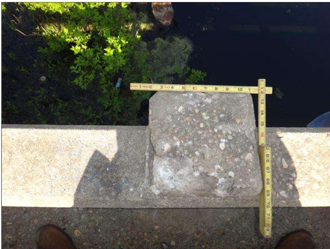
Span 2 Left Bridge Rail: top face at rail post 2, spall/delamination [8in x 8in x up to 1/4in deep]
