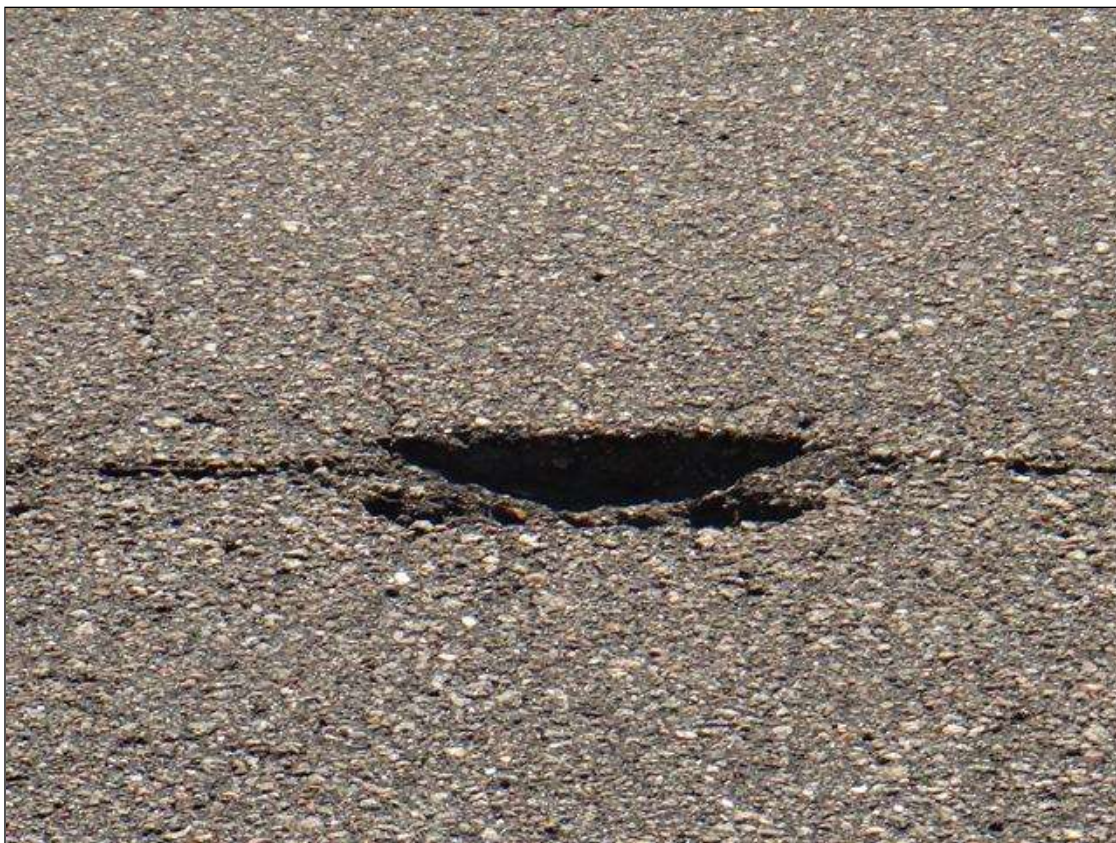
Span 1 Wearing Surface: centerline near midspan, pothole [11in x 5in x up to 2in deep]
