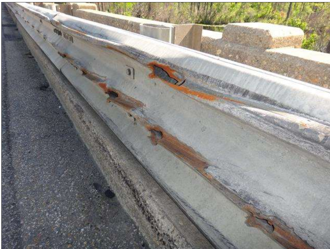
Span 1 Right Bridge Rail: along length of attached metal guardrail, vehicular impact damage with scrapes and tears [up to 12in x up to 3in]
