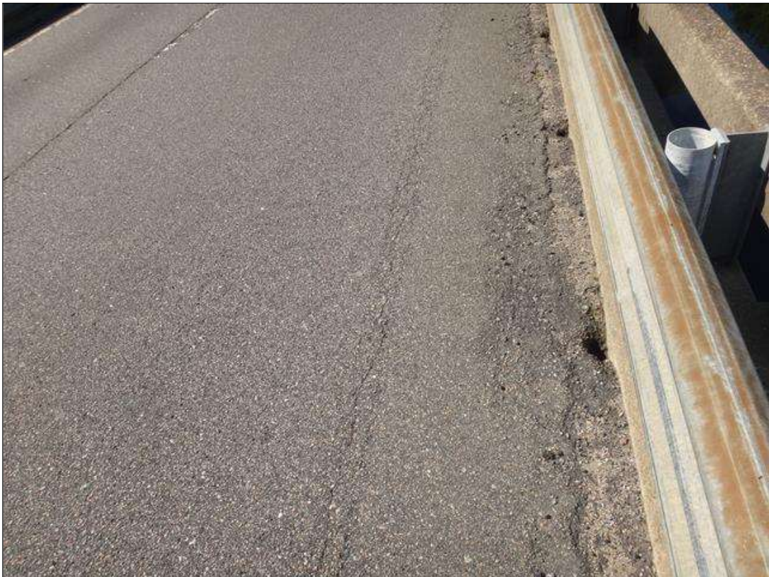
Span 4 Wearing Surface: 3ft from left shoulder, longitudinal crack [full length x up to 1/8in]
