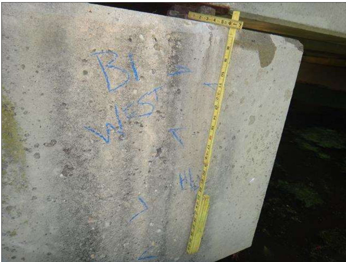
Bent 1 Cap 1: West face of cap, one [1] vertical crack [full height x hairline]
