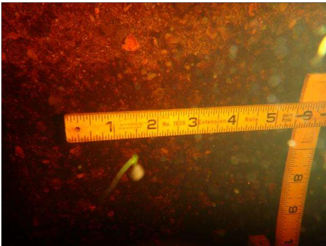
Bent 2 Pile 2: at waterline down 18in, minor abrasion [up to 1/16in deep]
