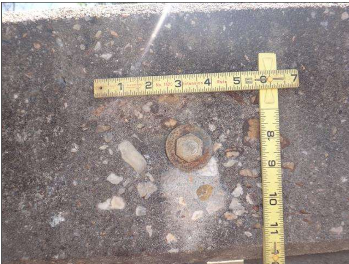
Span 4 Left Bridge Rail: along length of rail at steel rail connections, multiple spalls [up to 5in diameter x up to 1in deep]
