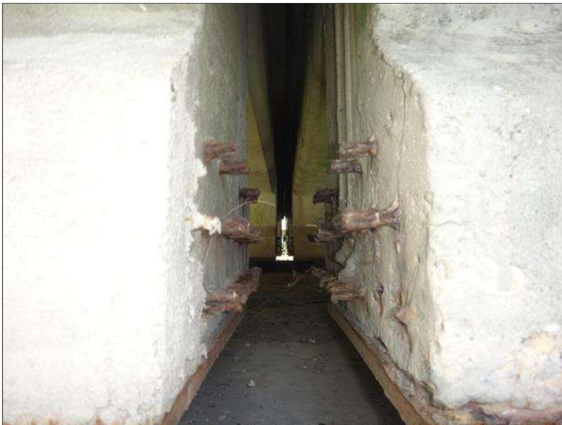
Exposed prestressing ends [similar at all beams at interior bents]
