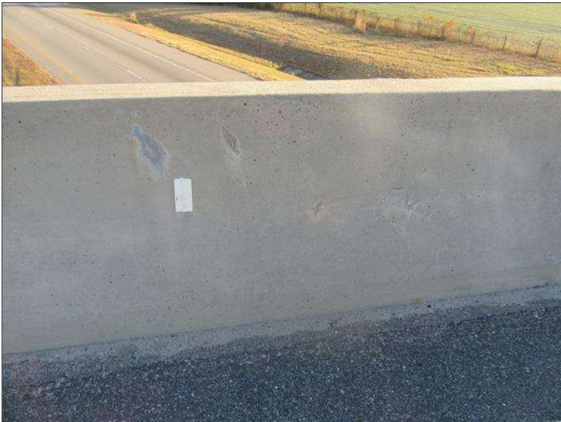
Span 4 Left Bridge Rail: HAIRLINE MAP CRACKING AT BENT 3
