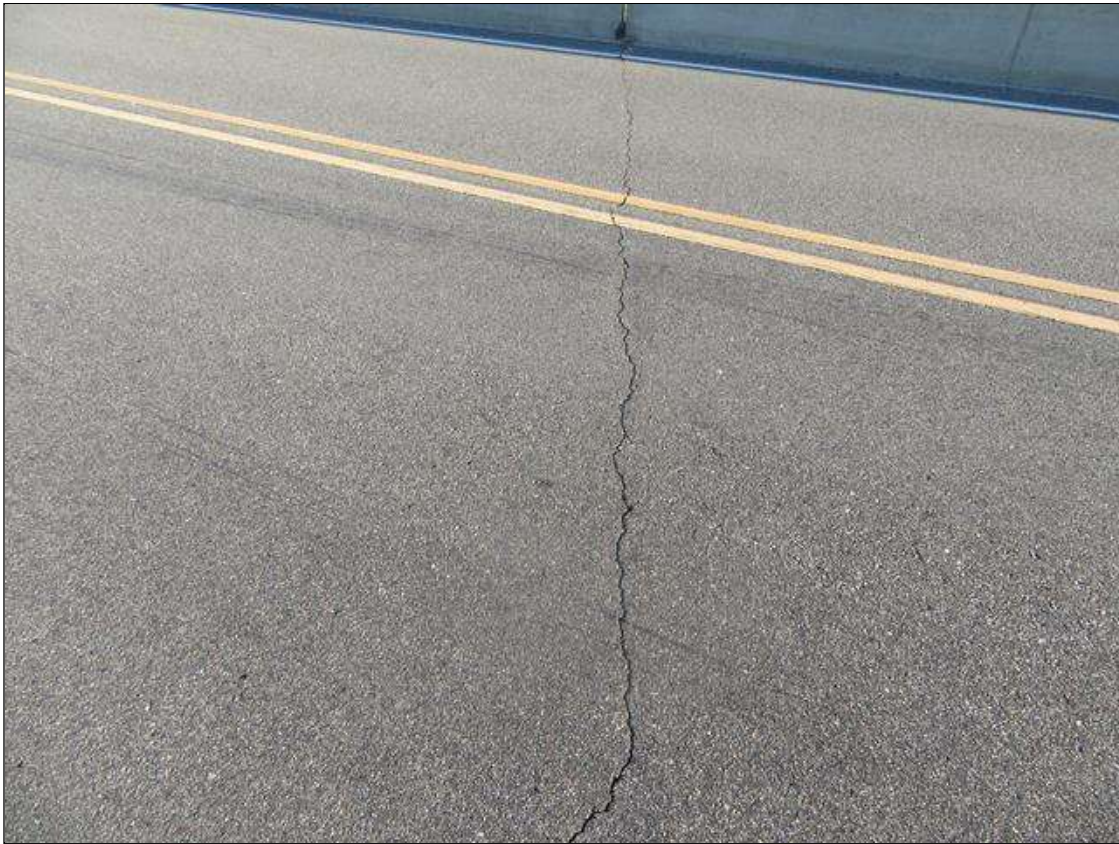
Span 4 Wearing Surface: 3/16" WIDE TRANSVERSE CRACK OVER BENT 3
