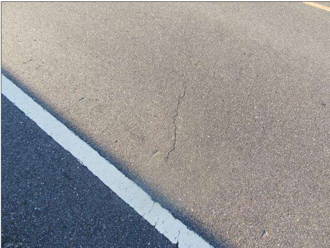
Span 1 Wearing Surface: 1/8" WIDE TRANSVERSE CRACK OVER END BENT 1 IN WESTBOUND LANE
