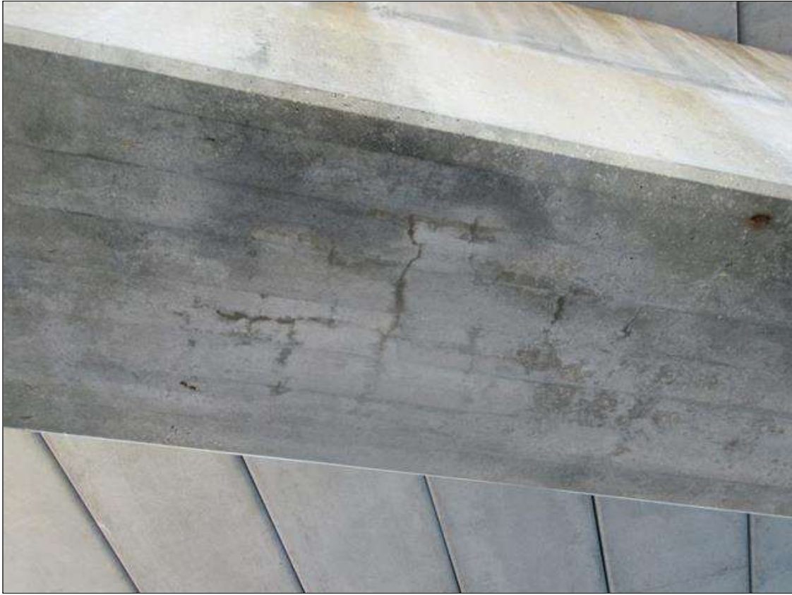
Bent 4 Cap 1: HAIRLINE TRANSVERSE CRACKS AT 1' SPACING IN BOTTOM OF CAP BETWEEN COLUMNS
