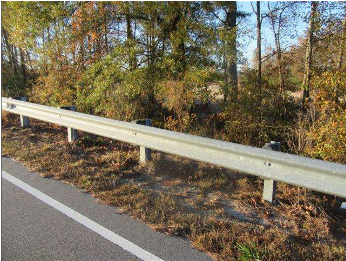
GUARDRAIL POST SPACING AT MID PORTION
