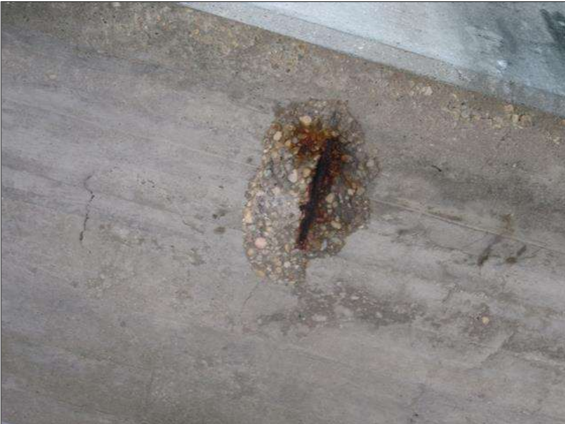
Bent 1 Cap 1: SPALL 14" LONG X 8" WIDE X 1.25" DEEP WITH 8" EXPOSED RUSTED REBAR. PRIORITY MAINTENANCE ISSUED
