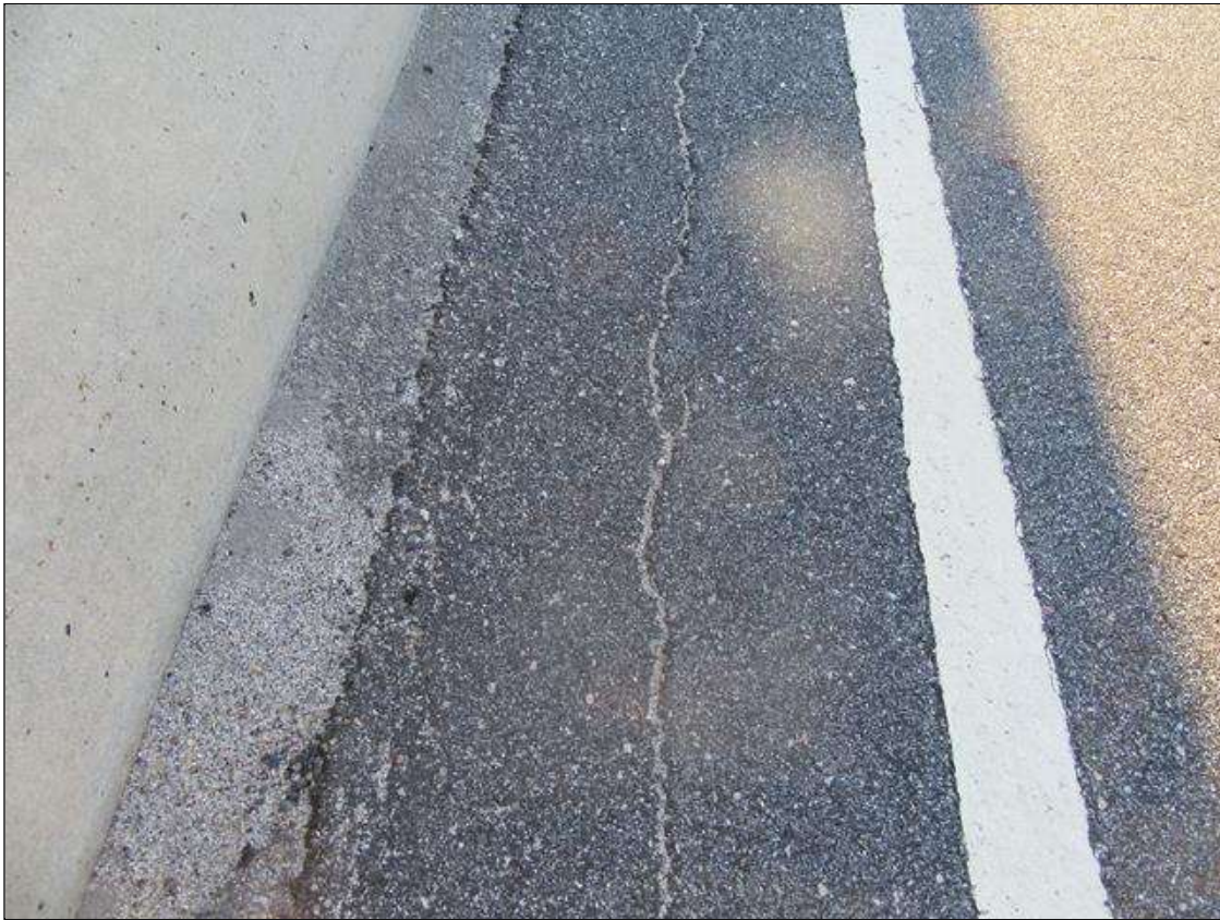
Span 3 Wearing Surface: 1/4" WIDE LONGITUDINAL CRACK IN LEFT SHOULDER AT BENT 2
