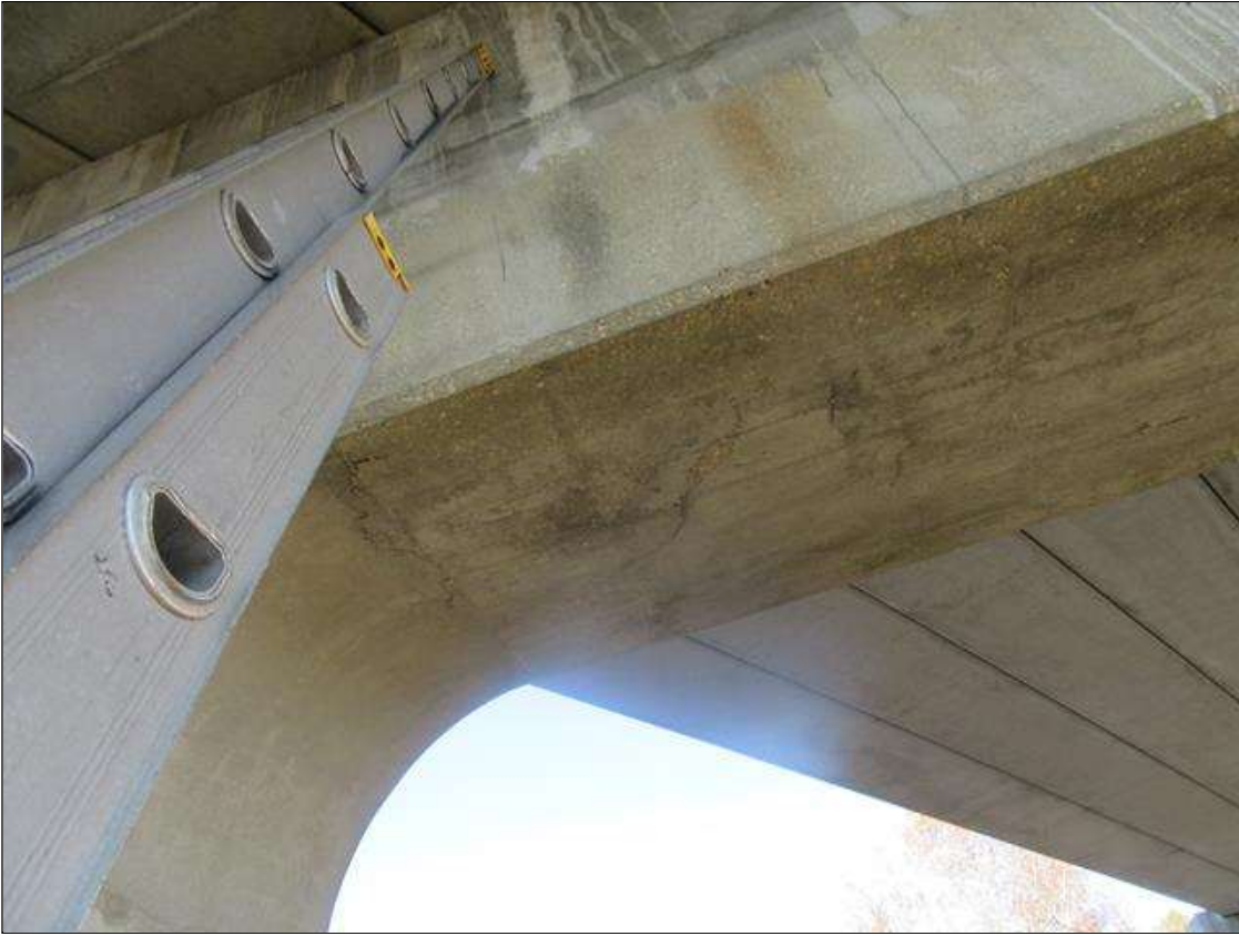
Bent 2 Cap 1: 2 FT. DIAMETER DELAMINATION IN BOTTOM OF CAP AT 2 FT. FROM COLUMN 2
