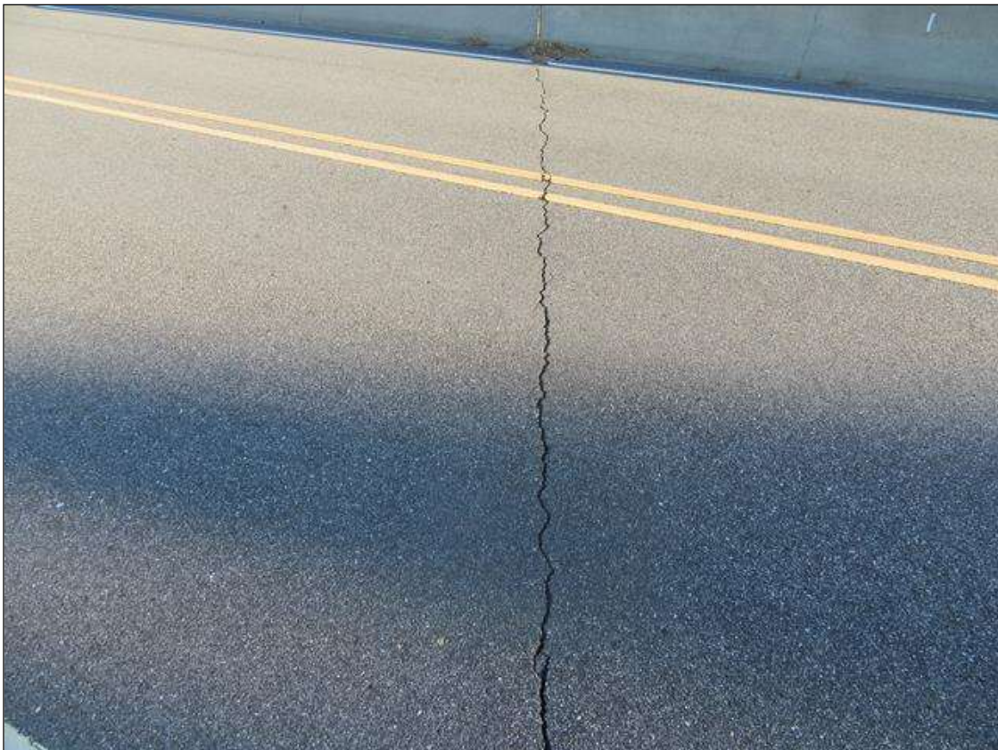
Span 5 Wearing Surface: 1/4" WIDE TRANSVERSE CRACK OVER BENT 4
