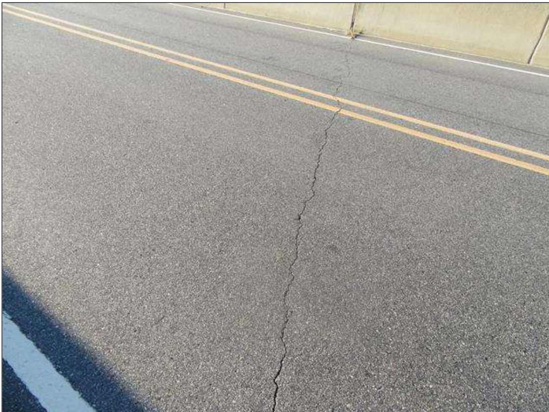
Span 3 Wearing Surface: 3/16" WIDE TRANSVERSE CRACK OVER BENT 2
