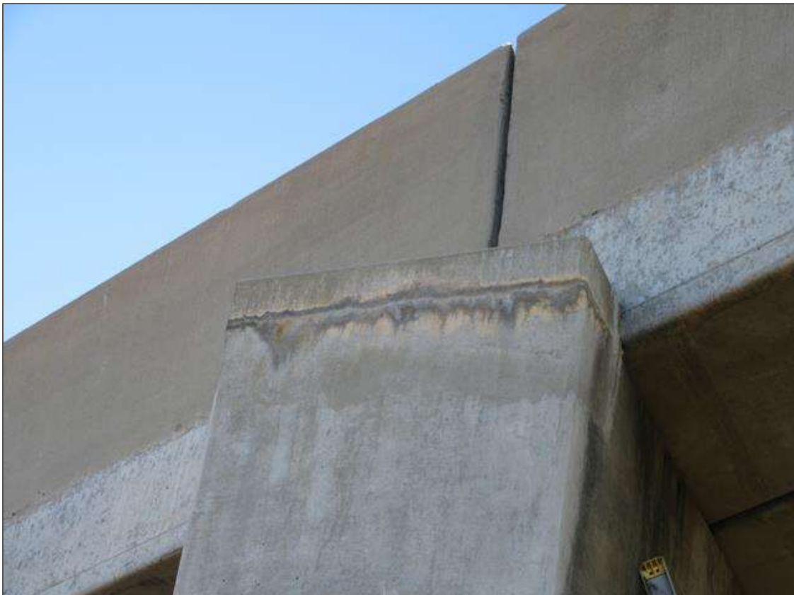
EFFLORESCENCE LEAKAGE AT BENT 2 LATERAL GUIDE
