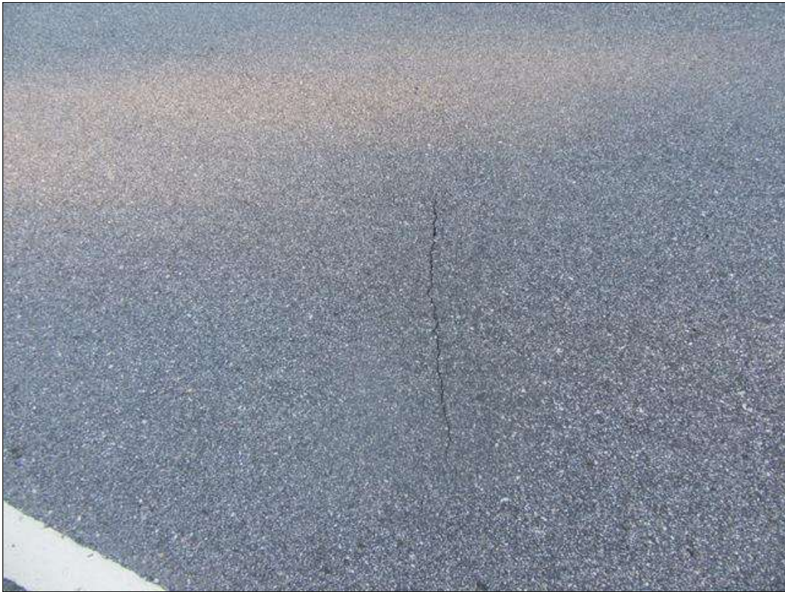
Span 5 Wearing Surface: 1/8" WIDE TRANSVERSE CRACK OVER END BENT 2
