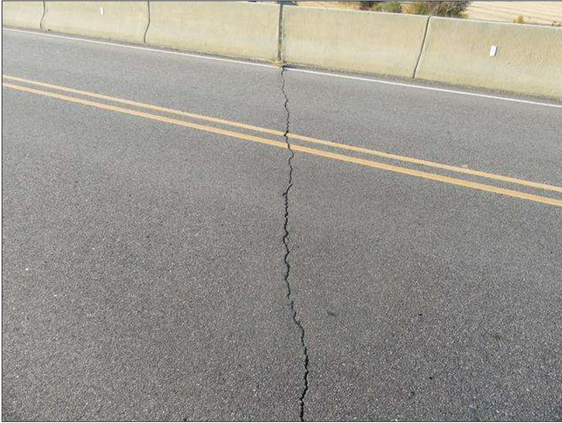
Span 2 Wearing Surface: 1/4" WIDE TRANSVERSE CRACK OVER BENT 1
