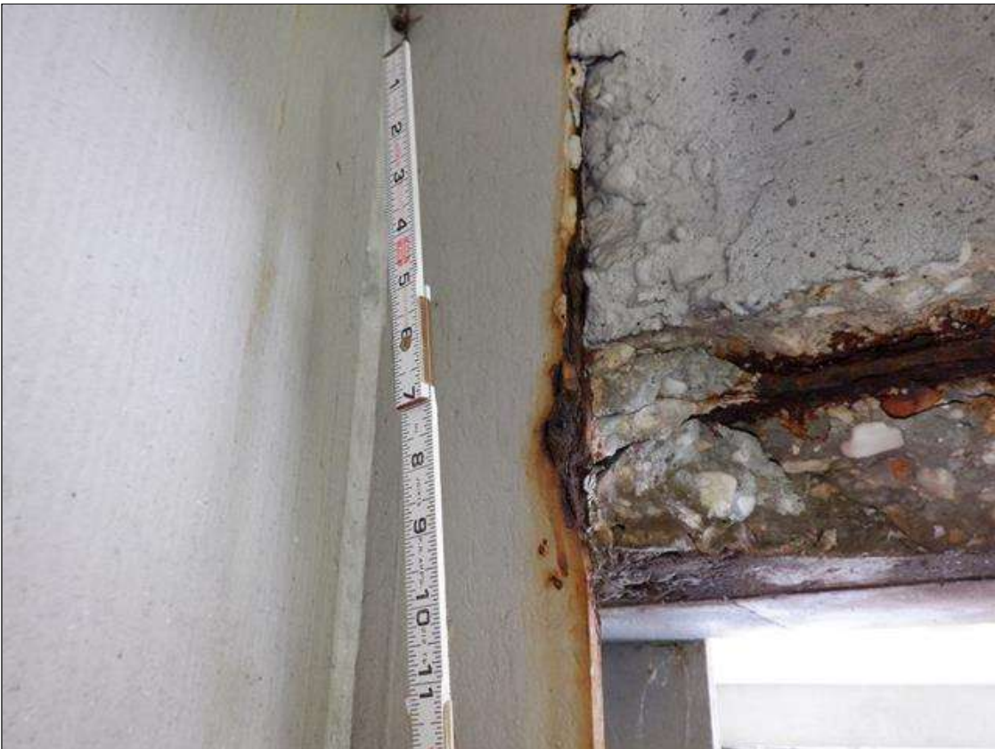
Span 3 Beam 3: 1 FT. OF CORROSION WITH 11/16" REMAINING SECTION IN WEB AROUND END DIAPHRAGM AND 1/4" REMAINING SECTION IN BEARING STIFFENER AT BENT 2 PAR
