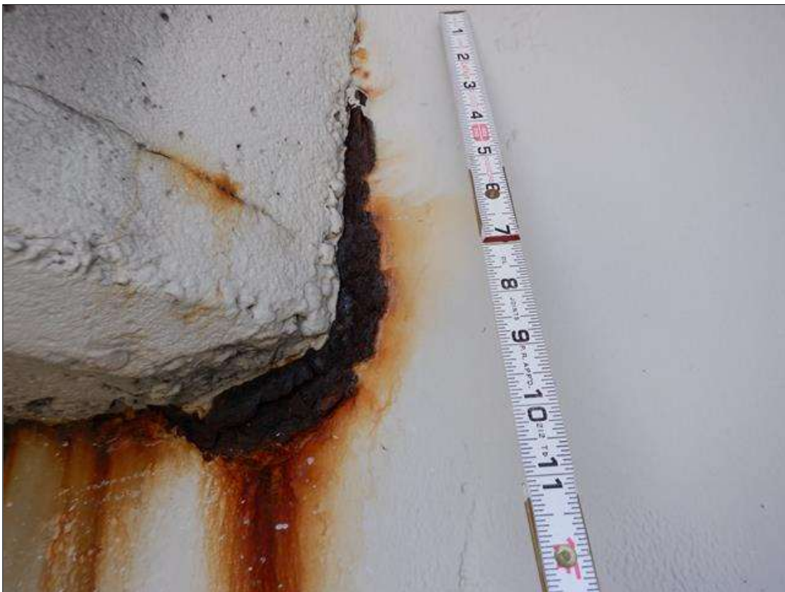
Span 2 Beam 1: 1 FT. OF CORROSION WITH 11/16" REMAINING SECTION IN WEB AROUND END DIAPHRAGM AT BENT 2 PAR
