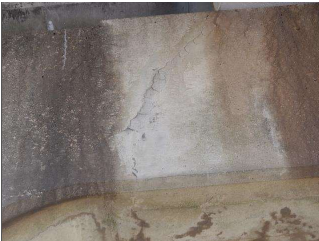
Bent 2 Cap 1: 3 FT. DIAGONAL HAIRLINE CRACK IN SOUTH FACE UNDER BAY 1
