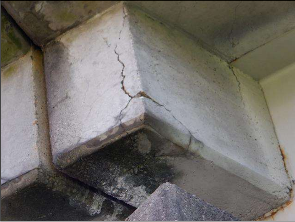
END DIAPHRAGM WEST OVERHANG AT BENT 1: 12" X 6" DELAMINATION IN SOUTH FACE
