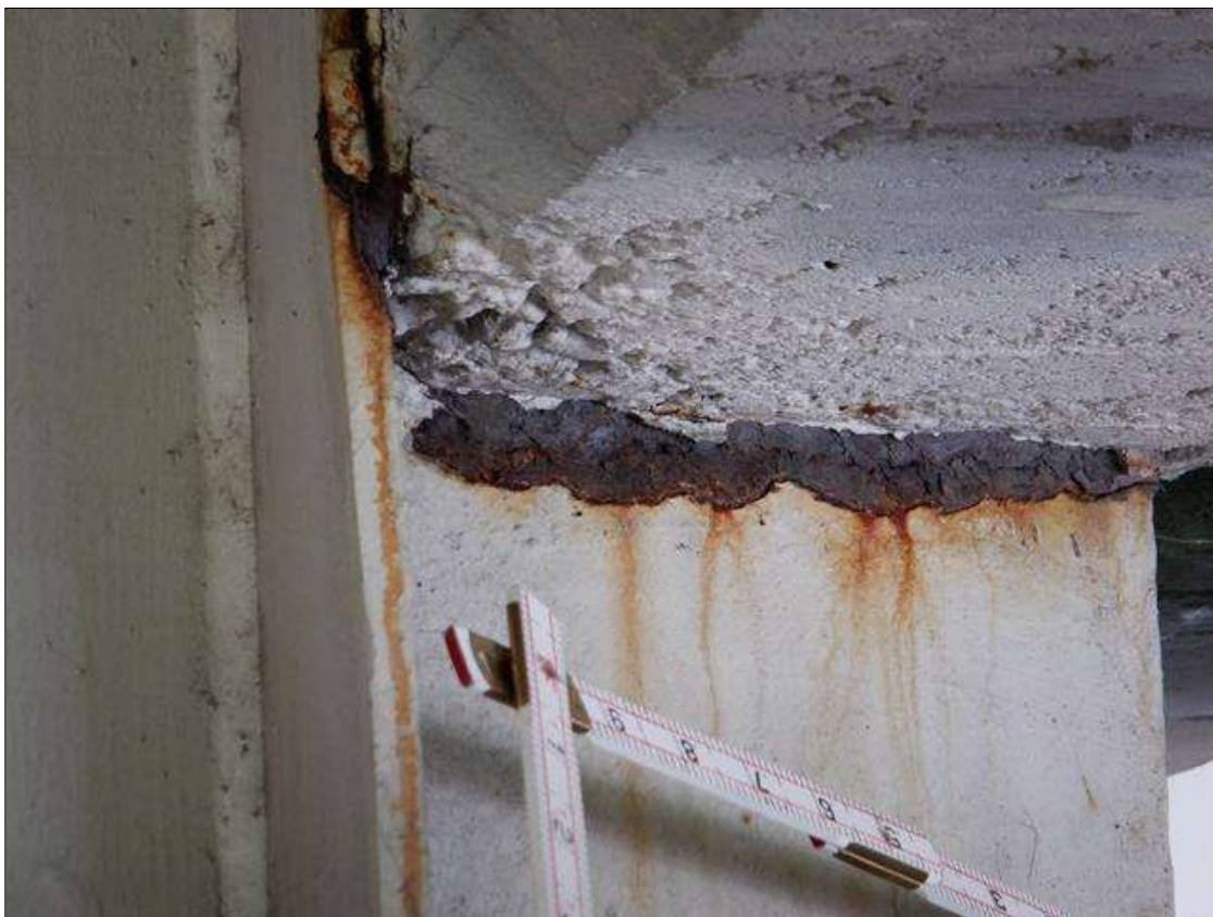
Span 1 Beam 2: 1 FT. OF CORROSION WITH 11/16" REMAINING SECTION IN WEB AROUND END DIAPHRAGM AT BENT 1 PAR
