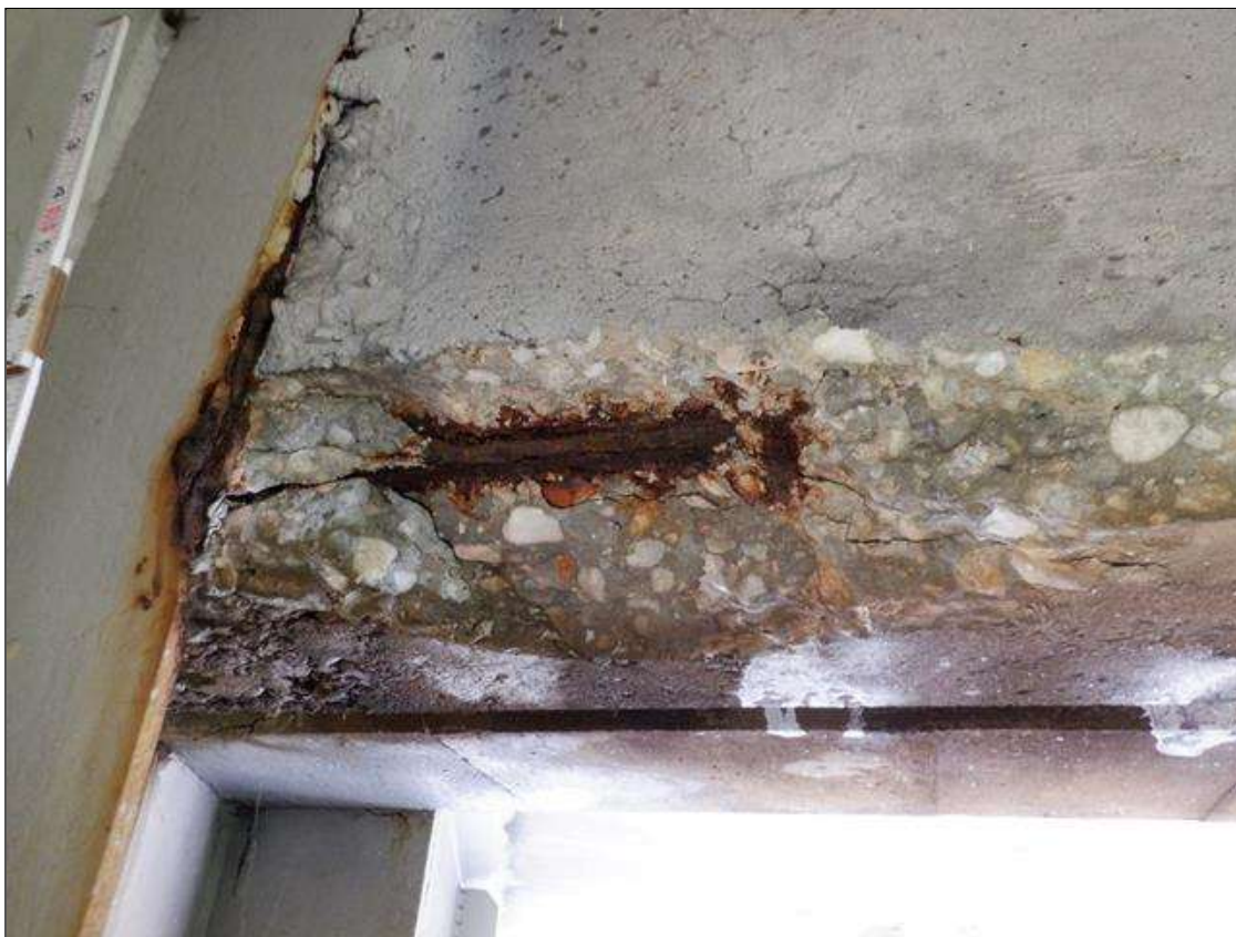
END DIAPHRAGM BAY 2 AT BENT 2: 12" X 3" X 2" DEEP SPALL WITH EXPOSED REBAR IN NORTH FACE PAR
