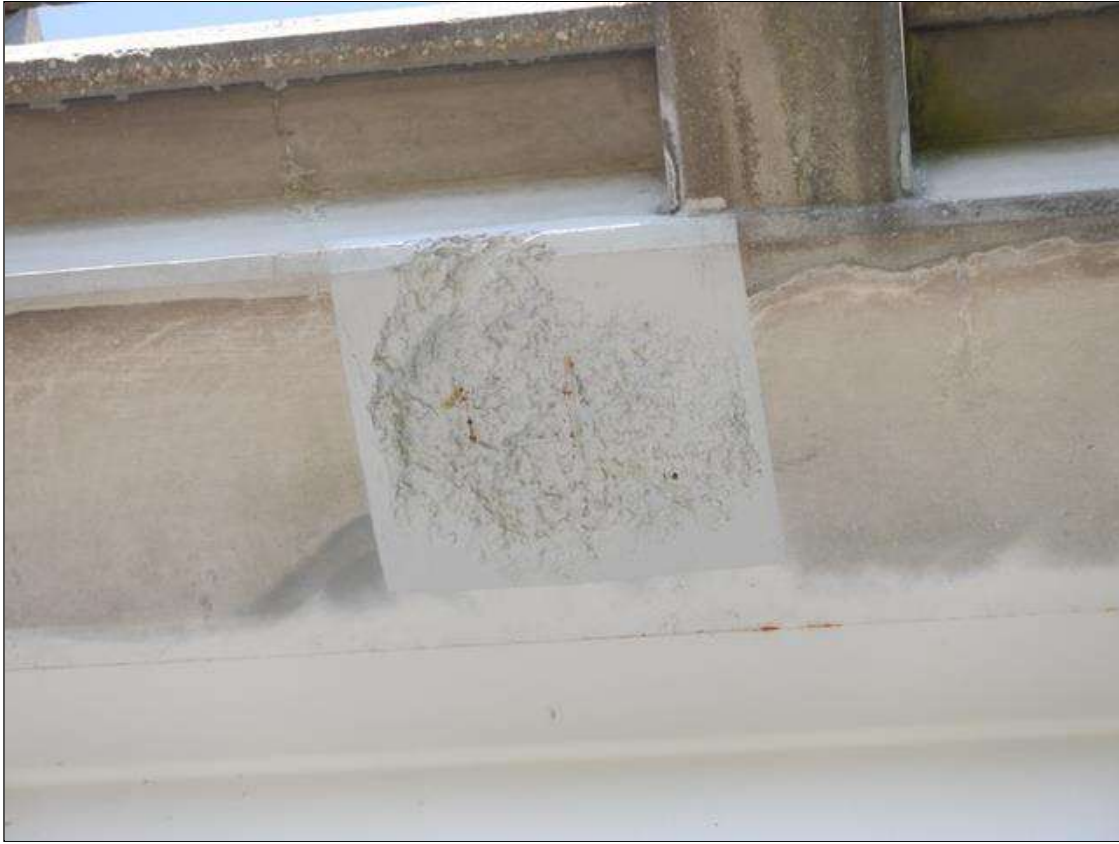
Span 2 Deck: 20" DIAMETER DELAMINATION IN BOTTOM OF DECK EAST OVERHANG 10 FT. FROM BENT 2. PAINTED OVER SPALL
