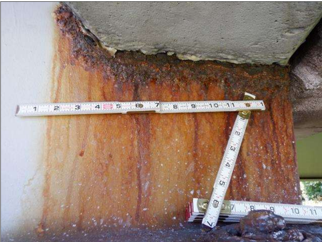
Span 2 Beam 1: 1 FT. OF CORROSION WITH 11/16" REMAINING SECTION IN WEB AROUND END DIAPHRAGM AT BENT 1 PAR
