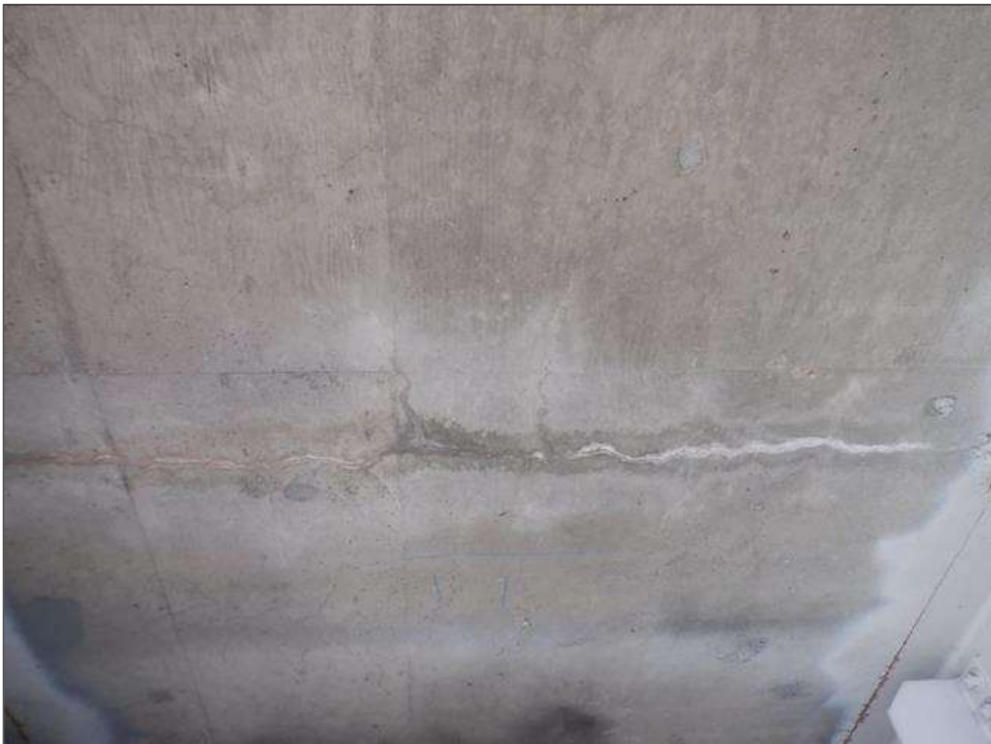
Span 1 Deck: 500 SF. OF HAIRLINE MAP AND TRANSVERSE CRACKING WITH EFFLORESCENCE IN BOTTOM OF DECK
