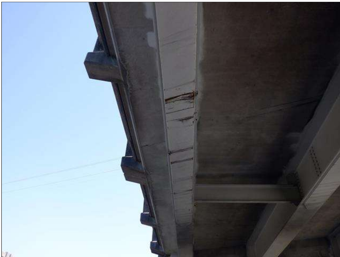
Span 2 Beam 1: 1 FT. OF VEHICLE SCRAPES IN BOTTOM FLANGE AND BOTTOM FLANGE COVER PLATE 25 FT. FROM BENT 1
