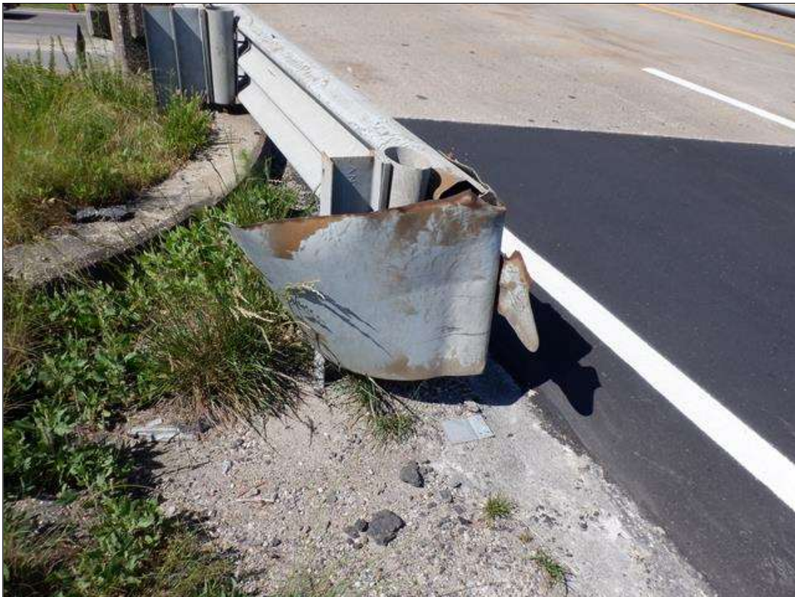
Span 3 Right Bridge Rail: IMPACT DAMAGE TO END OF BRIDGE RAIL PAR
