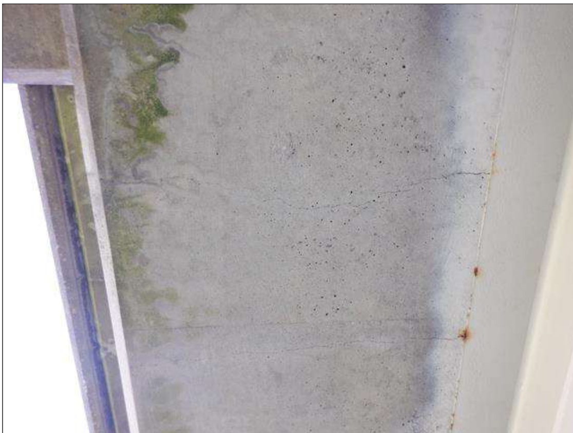
Span 1 Deck: 11 - 2 FT. TRANSVERSE HAIRLINE CRACKS WITH EFFLORESCENCE IN BOTTOM OF DECK WEST OVERHANG
