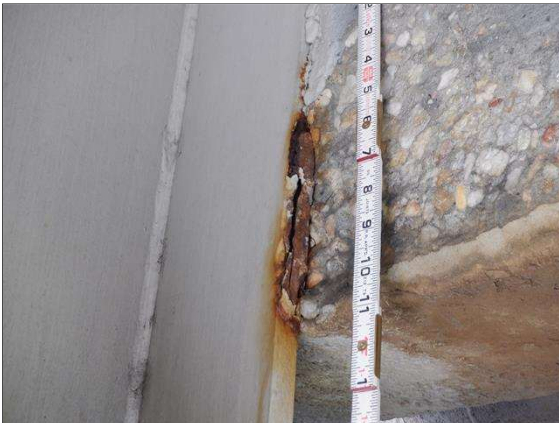
Span 2 Beam 4: 1 FT. OF CORROSION WITH 11/16" REMAINING SECTION IN WEB AROUND END DIAPHRAGM AT BENT 2 PAR
