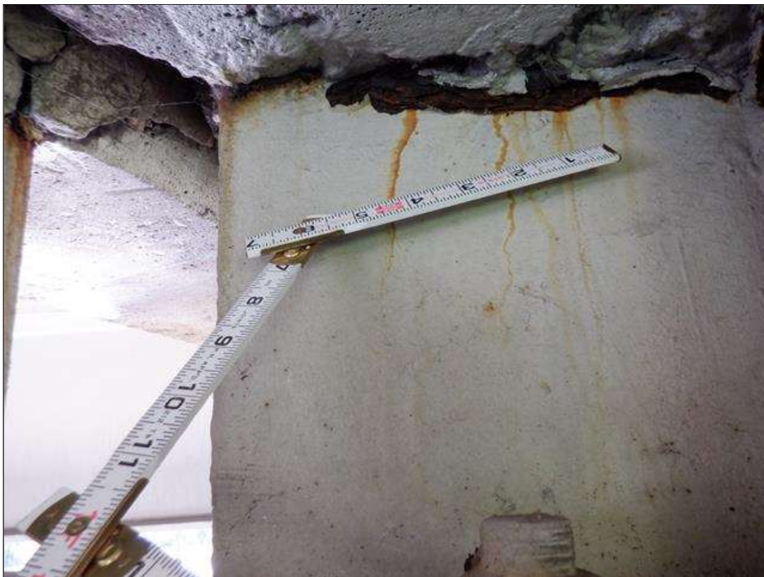
Span 1 Beam 3: 1 FT. OF CORROSION WITH 11/16" REMAINING SECTION IN WEB AROUND END DIAPHRAGM AT BENT 1 PAR
