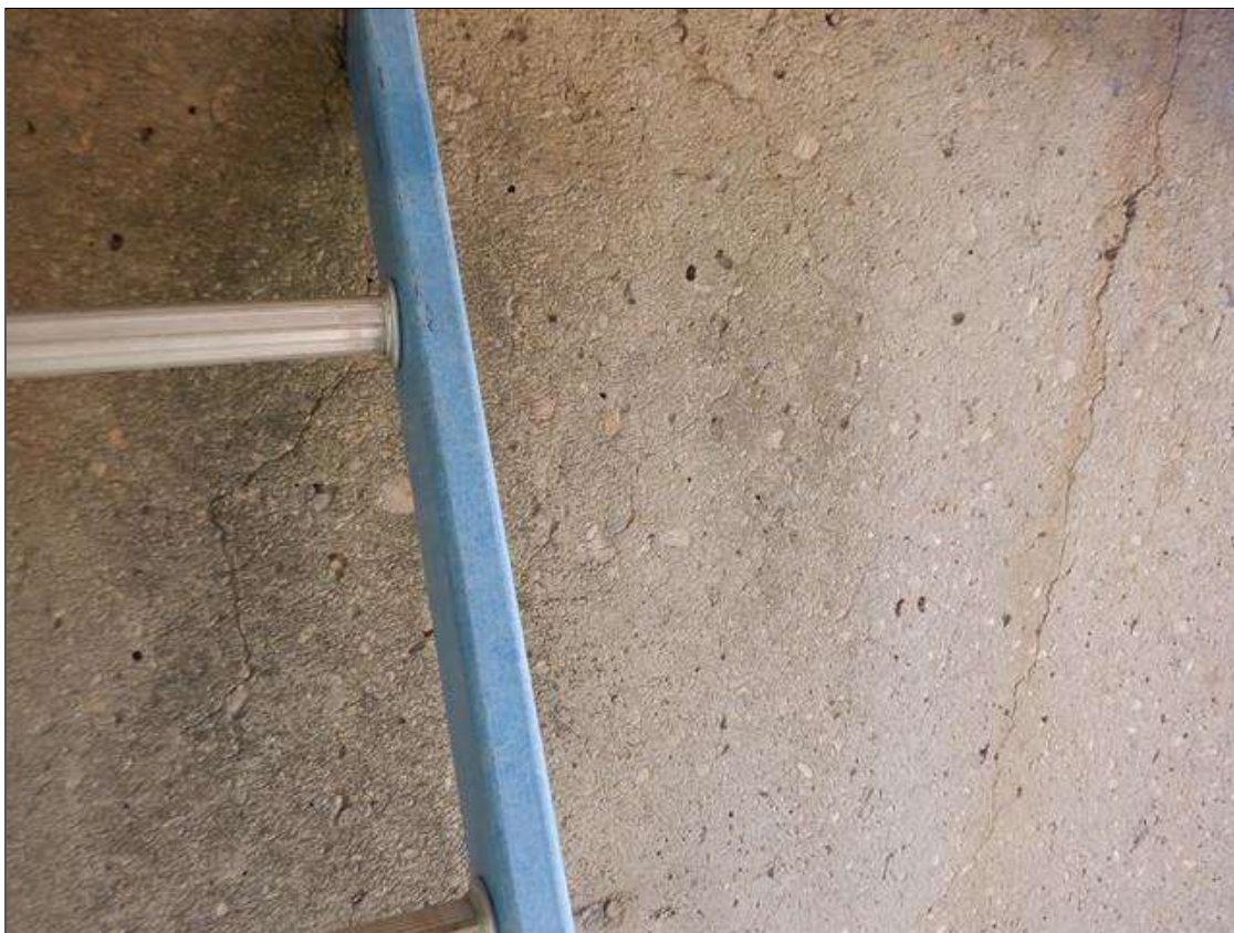
Bent 1 Cap 1: 2 - 36" VERTICAL HAIRLINE CRACKS IN SOUTH FACE UNDER BAY 3
