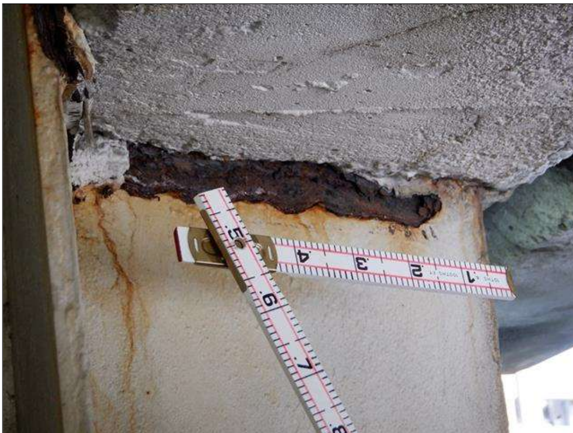
Span 1 Beam 1: 1 FT. OF CORROSION WITH 11/16" REMAINING SECTION IN WEB AROUND END DIAPHRAGM AT BENT 1 PAR
