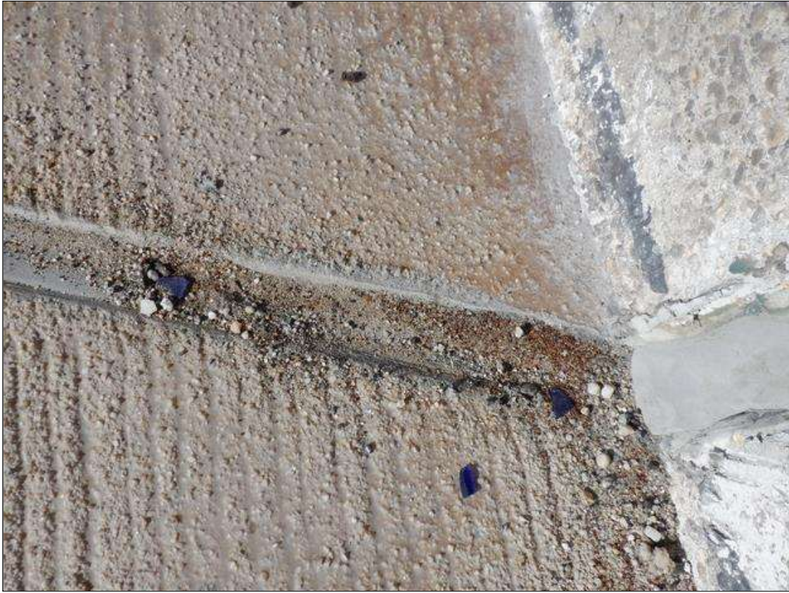
Expansion Joint : 3FT OF DEBRIS IMPACTION
