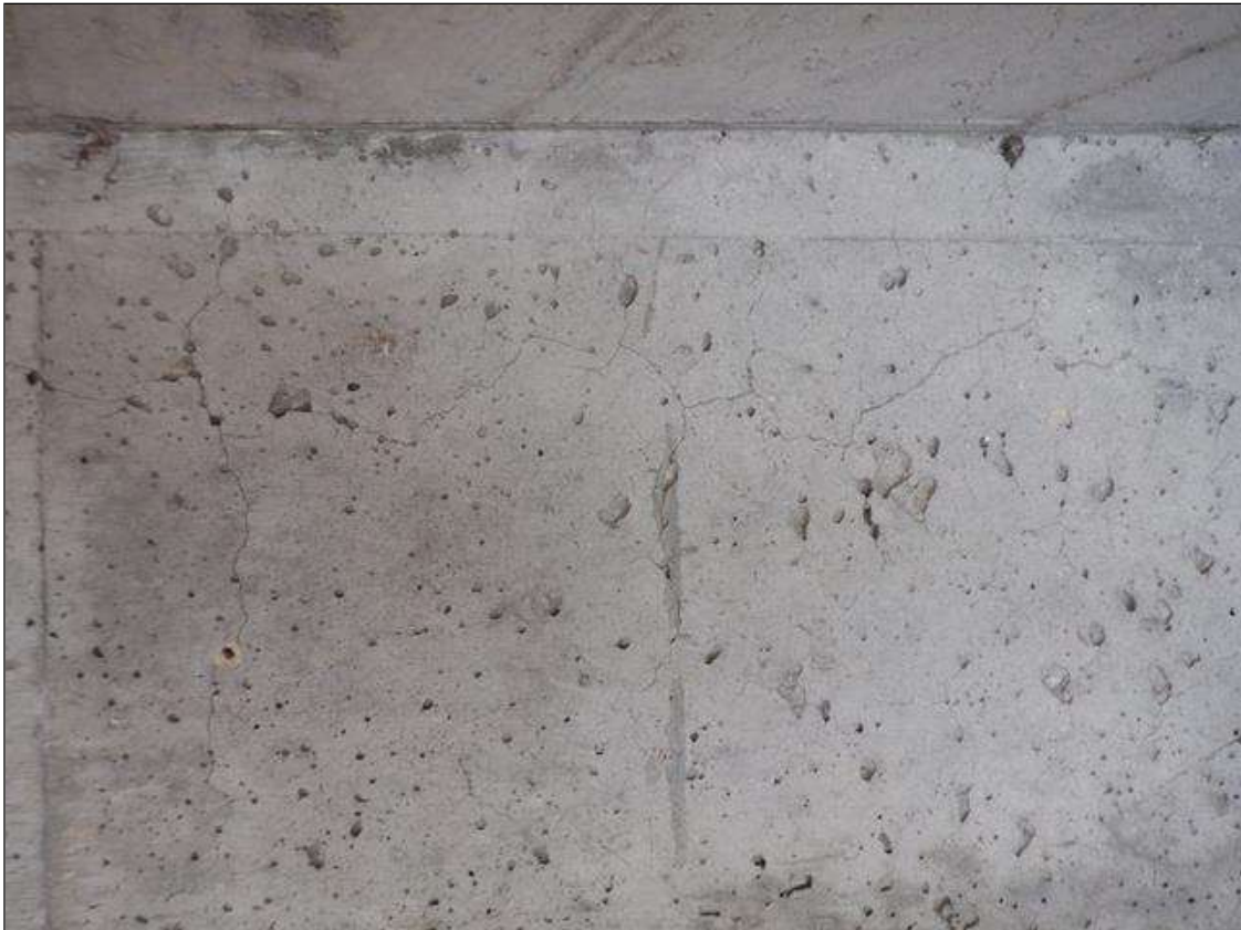
End Bent 1 Abutment/Backwall : 8 SF. OF HAIRLINE MAP CRACKING IN BAY 3
