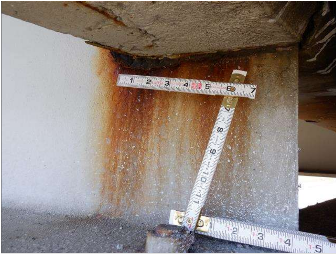
Span 2 Beam 4: 1 FT. OF CORROSION WITH 11/16" REMAINING SECTION IN WEB AROUND END DIAPHRAGM AT BENT 2 PAR
