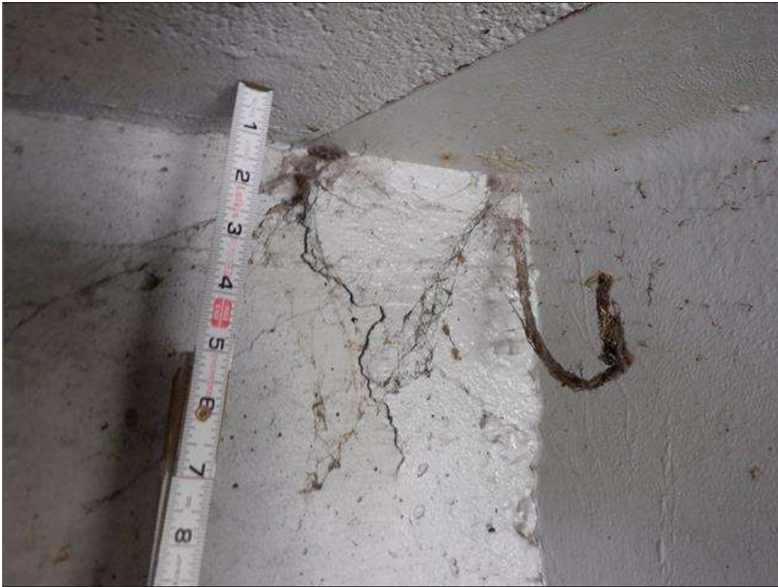
End Bent 1 Abutment/Backwall : 6" X 4" DELAMINATION IN BAY 2
