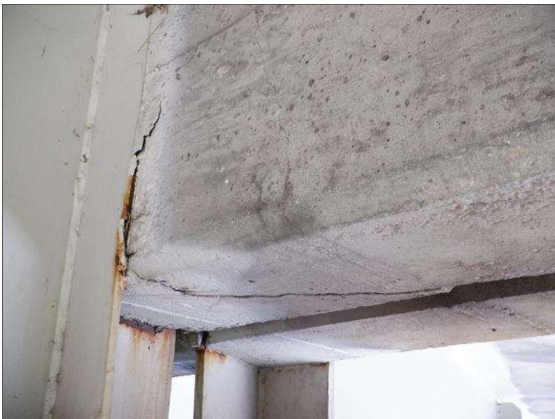
END DIAPHRAGM BAY 3 AT BENT 1: 18" X 6" DELAMINATION IN SOUTH FACE
