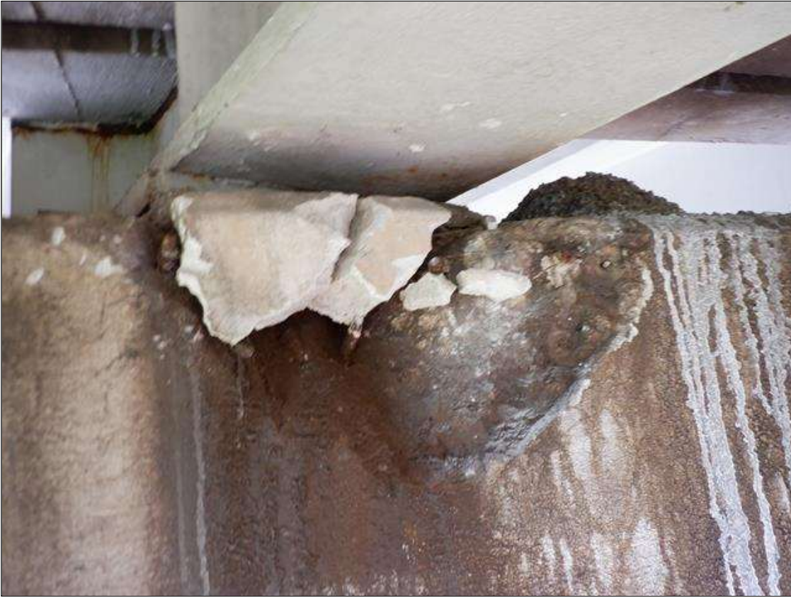
Bent 2 Cap 1: 18" X 6" X 4" FAILED PATCH WITH 4" X 1 1/2" LOSS OF BEARING AREA IN NORTH FACE UNDER BEAM 3 PAR
