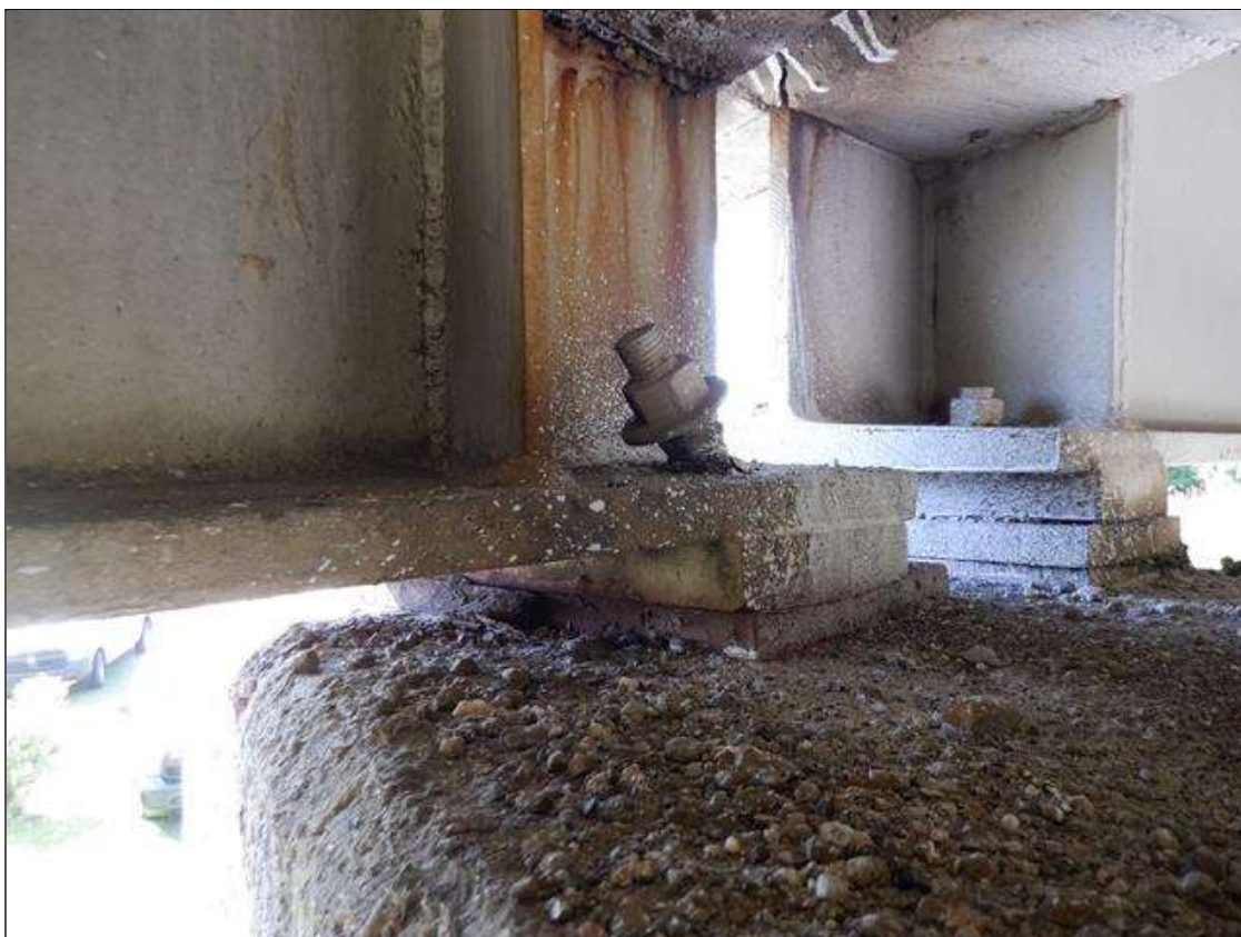
Span 3 Beam 4 Near Bearing: EAST AND WEST ANCHOR BOLT LEANING TOWARDS NORTH PAR
