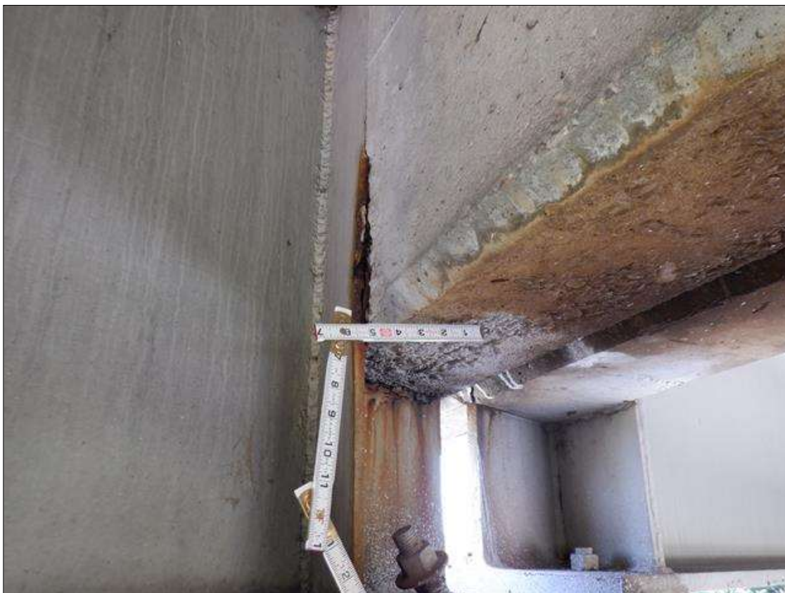
Span 3 Beam 4: 1 FT. OF PAINTED OVER PITTING UP TO 1/16" DEEP WITH RUST BLEEDING IN WEB AROUND END DIAPHRAGM AT BENT 2
