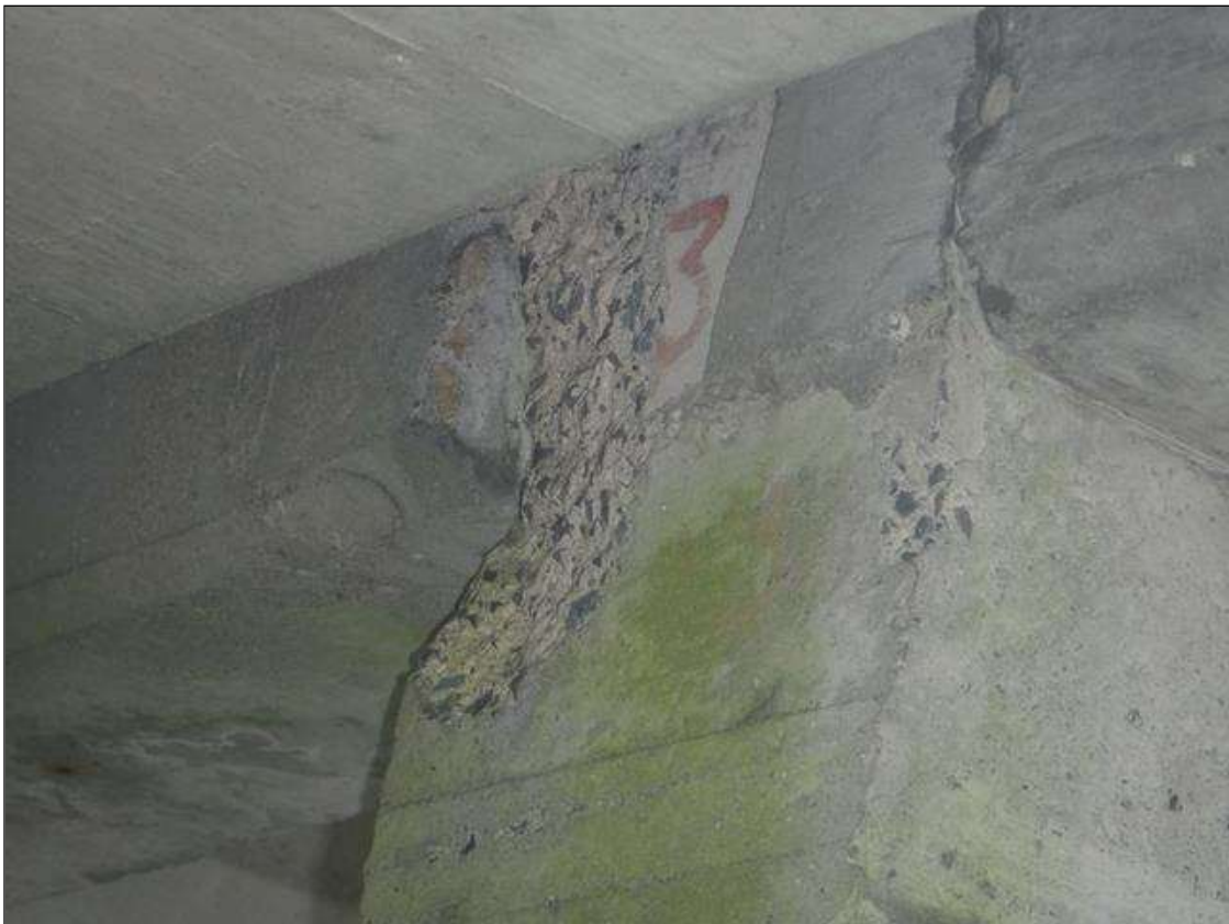
Span 2 Beam 4: 14" X 7" X 2" DEEP SPALL IN END OF BEAM AT BENT 1
