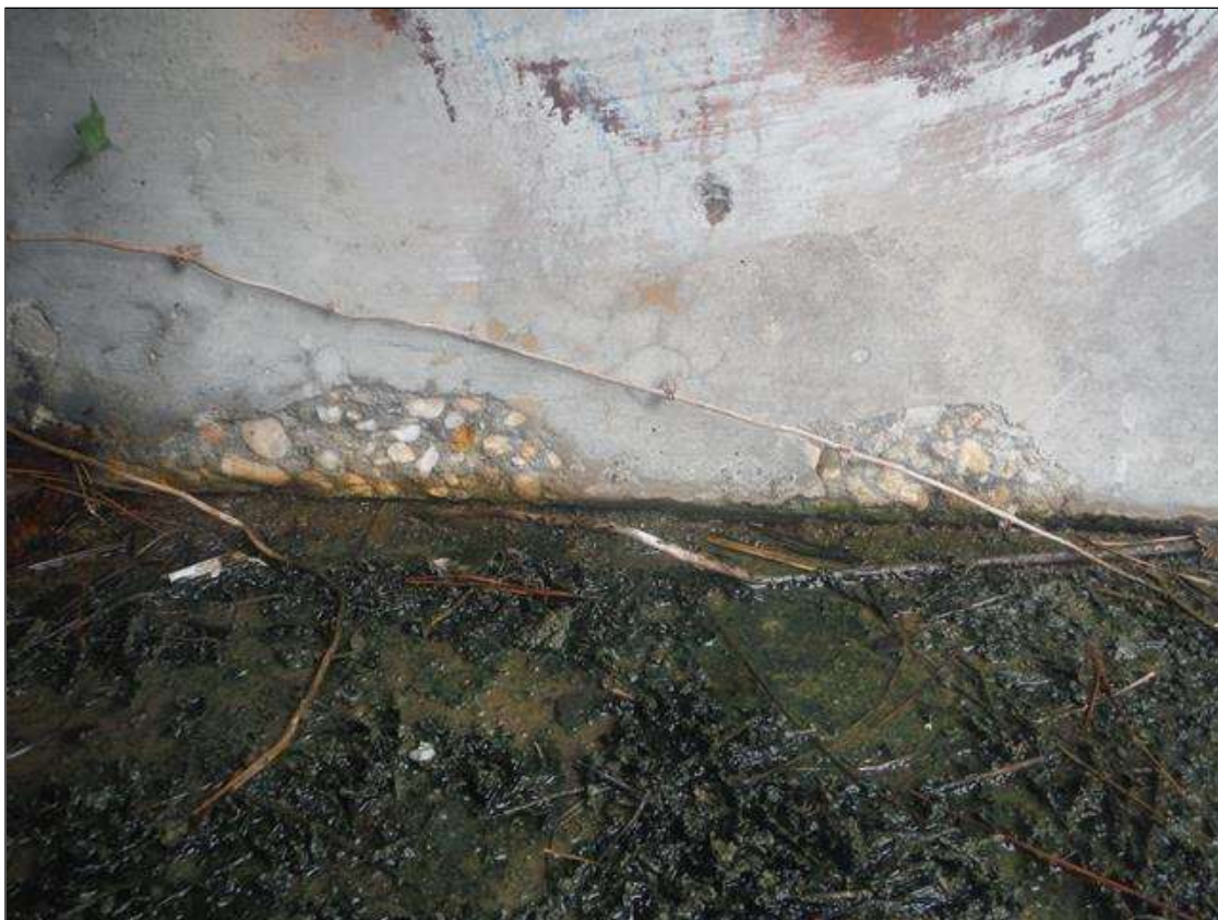
End Bent 1 Abutment/Backwall : 2 - SPALLS UP TO 12" X 4" X 1/2" DEEP AT NORTH END
