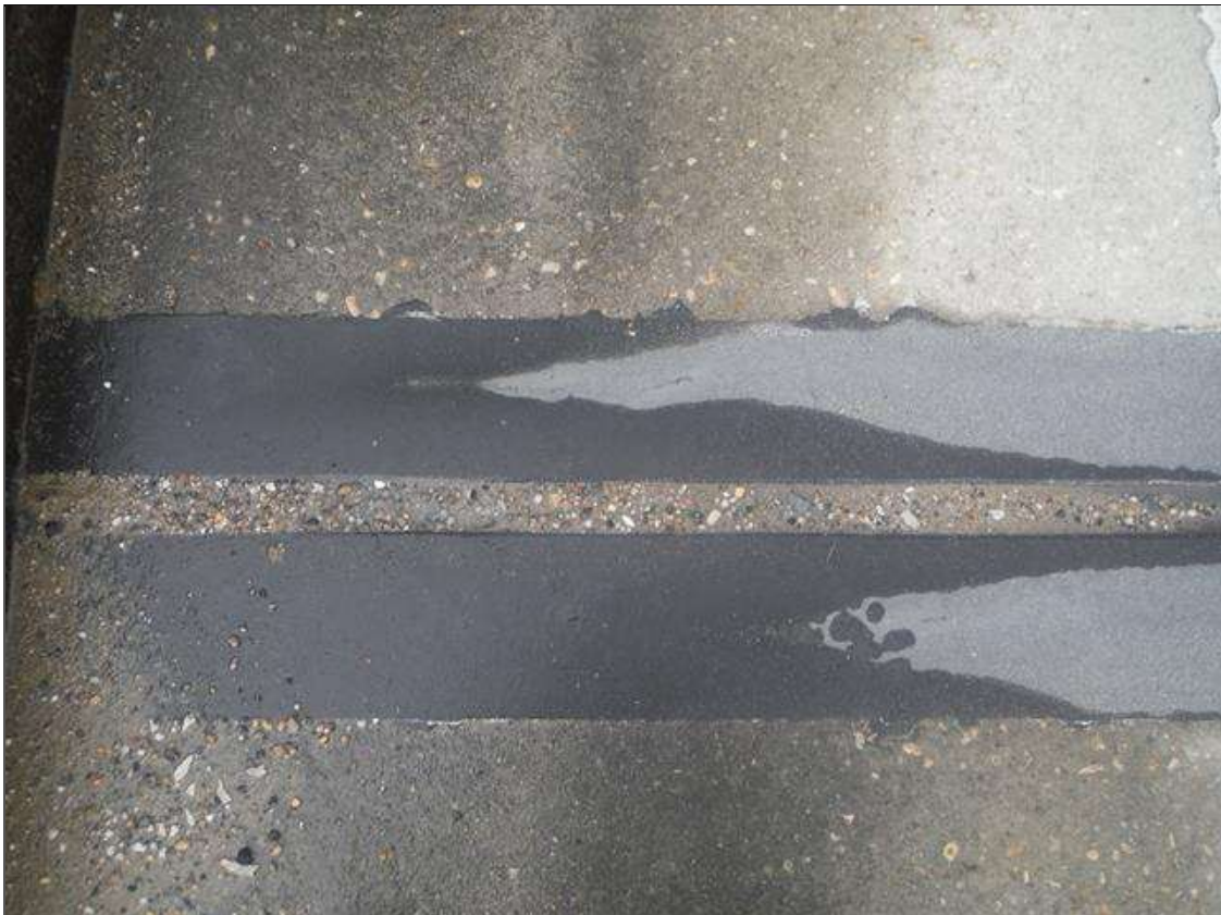
Expansion Joint : 6 FT. OF DEBRIS IMPACTION
