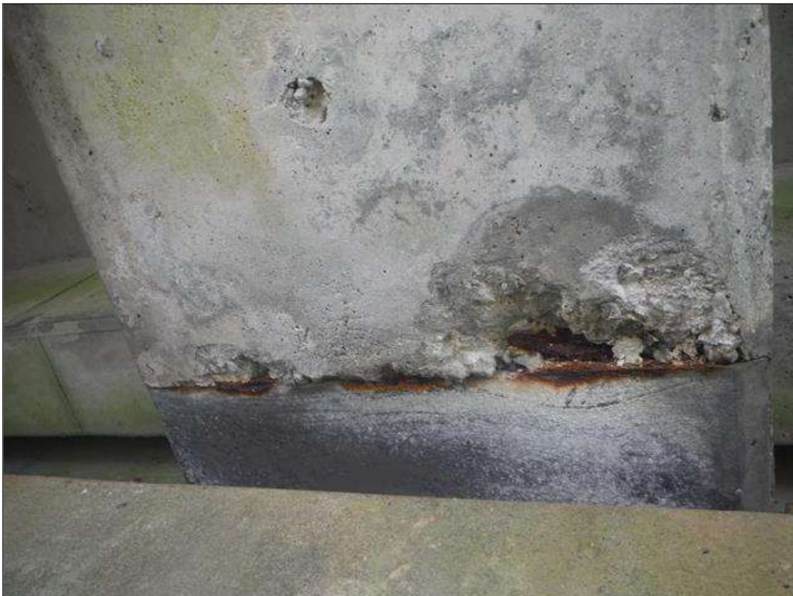
Span 2 Beam 3: 3" X 7" X 1/2" DEEP SPALL WITH EXPOSED REBAR IN BOTTOM FACE AT BENT 2
