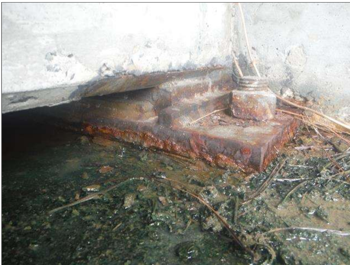
Span 1 Beam 1 Near Bearing: SURFACE CORROSION
