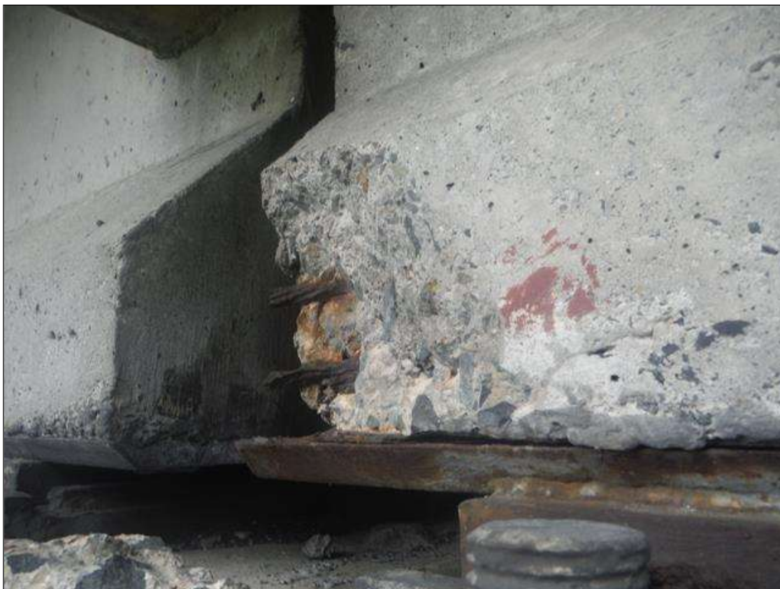
Span 1 Beam 1: 7" X 5" X 2" DEEP SPALL WITH EXPOSED STRANDS IN BOTTOM FLANGE NORTH FACE AT BENT 1 (PM)
