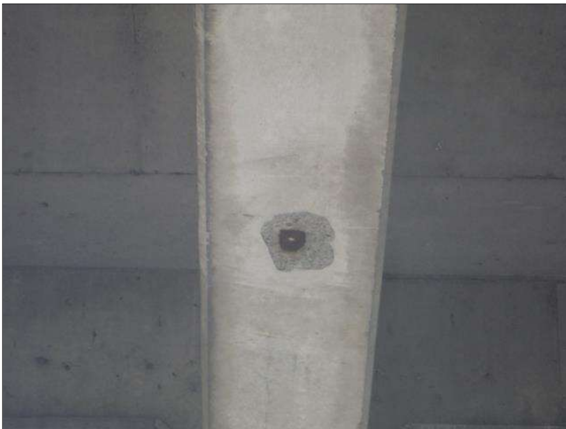
Span 3 Beam 4: 10" DIAMETER X 1/2" DEEP SPALL IN BOTTOM FACE AT TIE-DOWN POINT NEAR MIDSPAN
