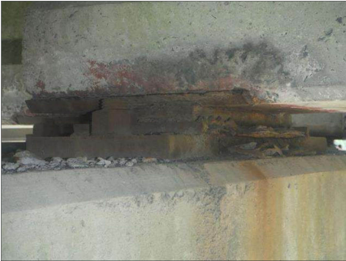
Span 1 Beam 3 Far Bearing: 1/4" OF PACK RUST
