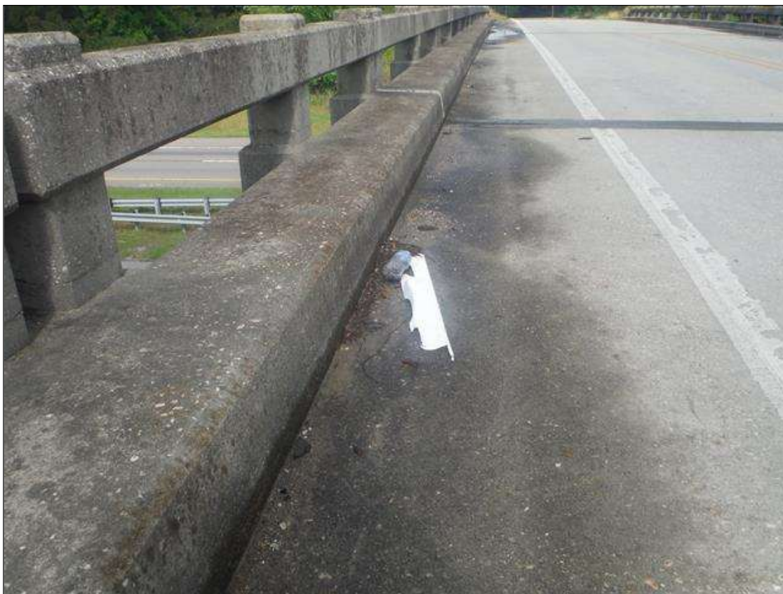
DEBRIS ALONG SOUTH CURB
