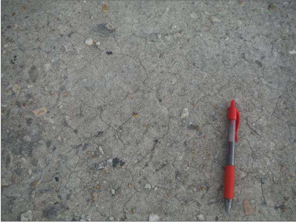
Span 1 Deck: 1376 SF. OF HAIRLINE MAP CRACKING AND TRANSVERSE AND DIAGONAL CRACKING UP TO 1/16" WIDE IN TOP OF DECK
