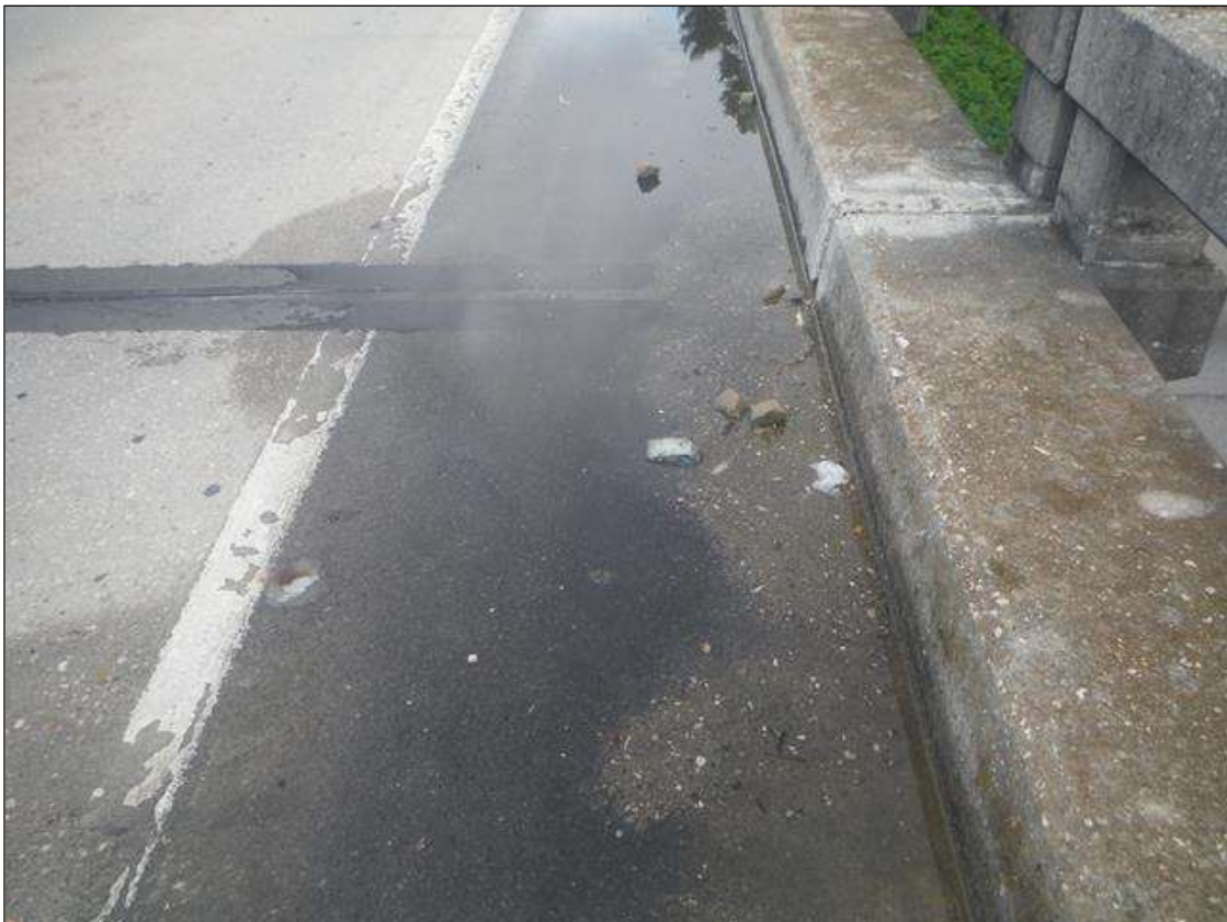
PONDING WATER ALONG NORTH AND SOUTH CURB
