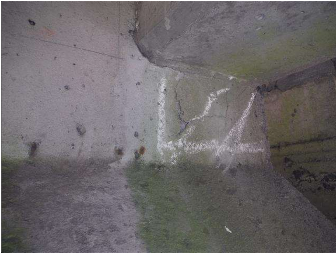
Span 2 Beam 3: 7" X 3" DELAMINATION IN WEB SOUTH FACE AT BENT 2
