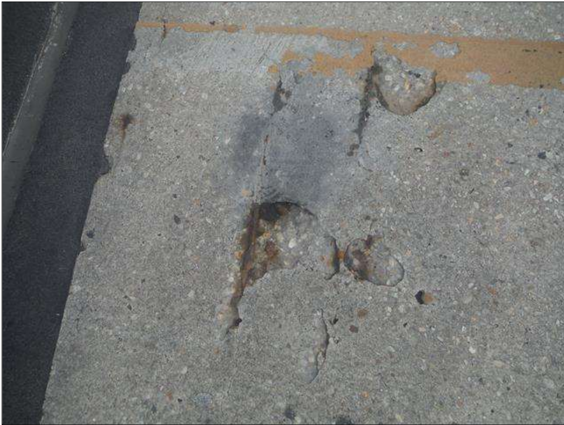
Span 2 Deck: 20" X 12" X 1/2" DEEP SPALL WITH EXPOSED REBAR IN TOP OF DECK AT BENT 1
