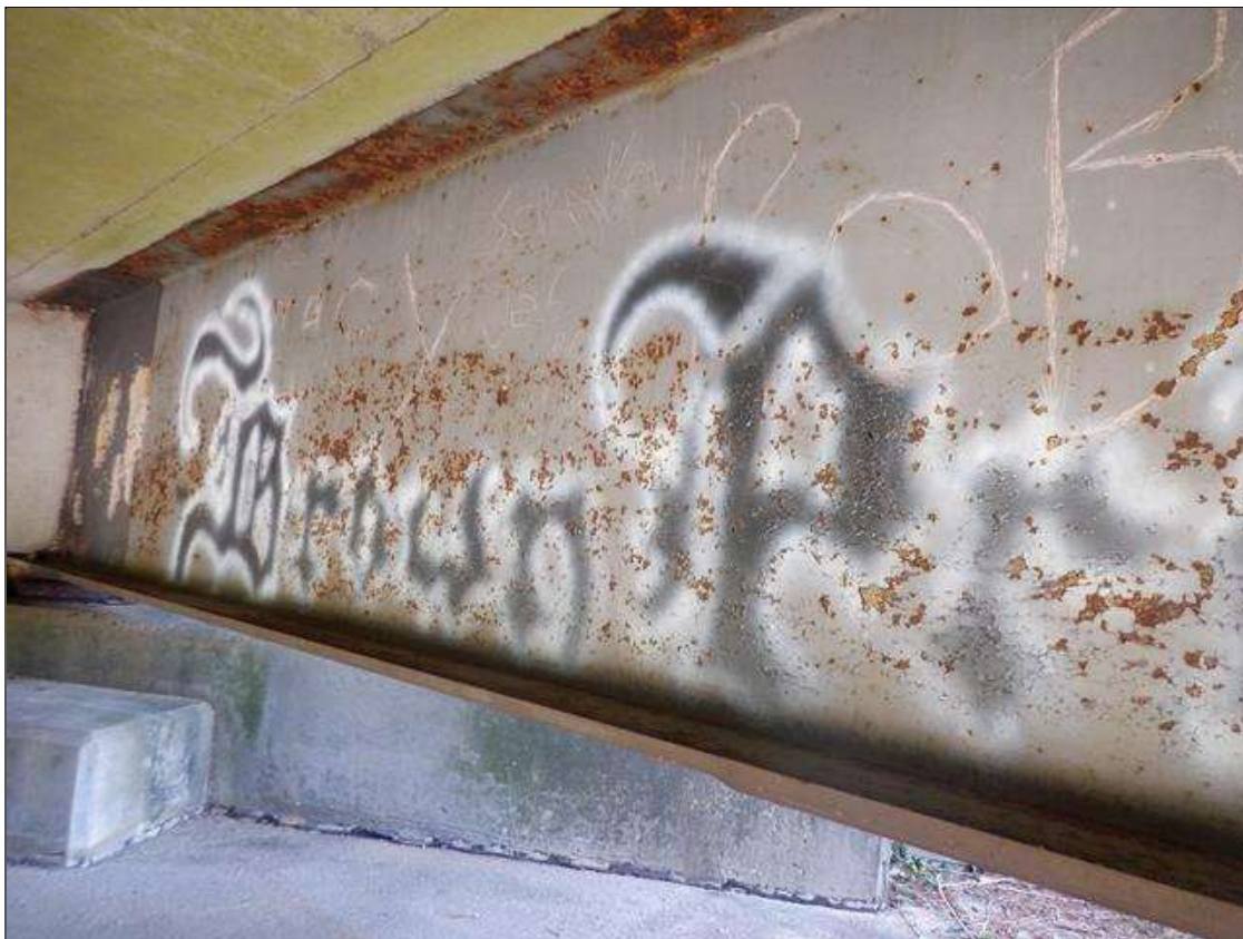
Span 1 Beam 1: PAINT PEELING WITH SURFACE RUST , NO SECTION LOSS
