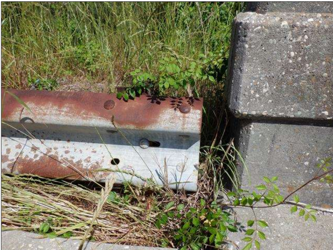
NW GUARDRAIL NOT ATTACHED. OTHER LOCATIONS SIMILAR
