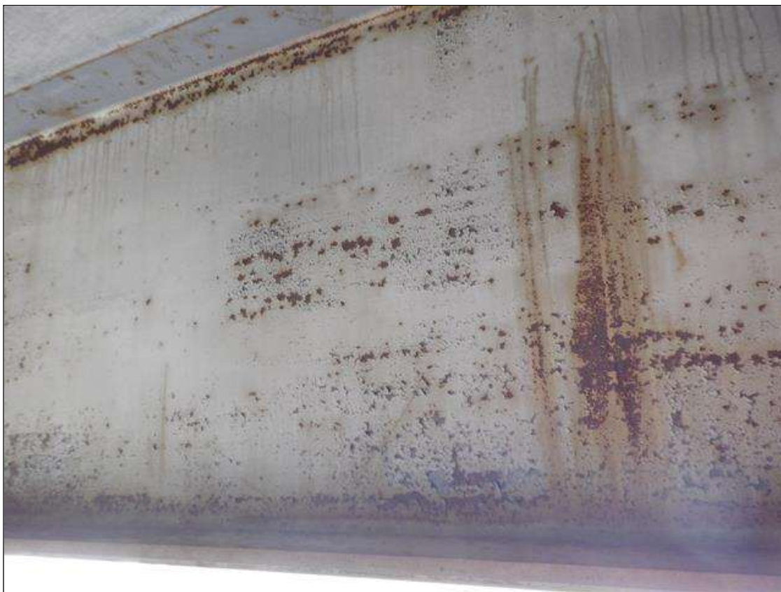
Span 5 Beam 2: PAINT PEELING AND SURFACE RUST IN FLANGES AND WEBS
