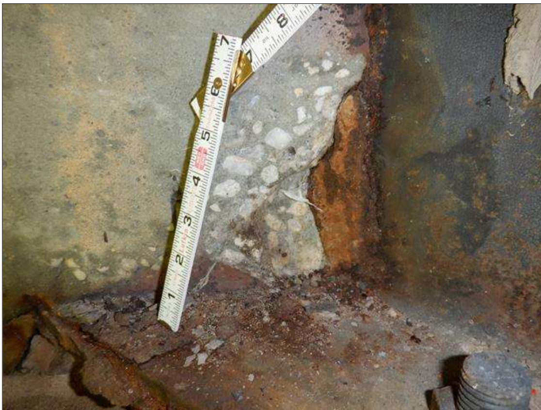
End Bent 1 Abutment/Backwall : SPALL MEASURING 7" HIGH X 4" WIDE X 1" DEEP LOCATED BAY 3 ADJACENT TO BEAM 3
