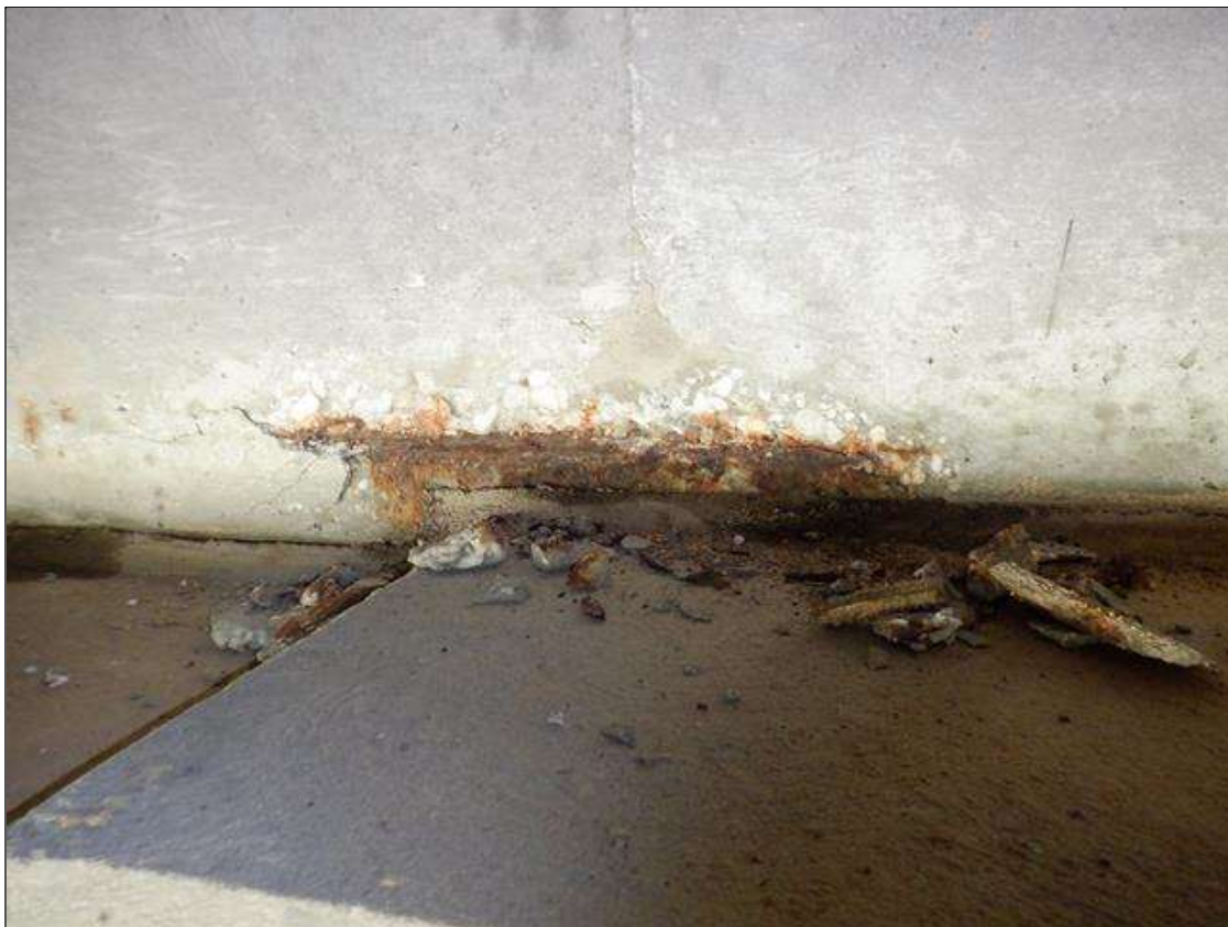
End Bent 2 Abutment/Backwall : SPALL 1.5 FT LONG X 4" WIDE X 1" DEEP LOCATED IN BAY 2
