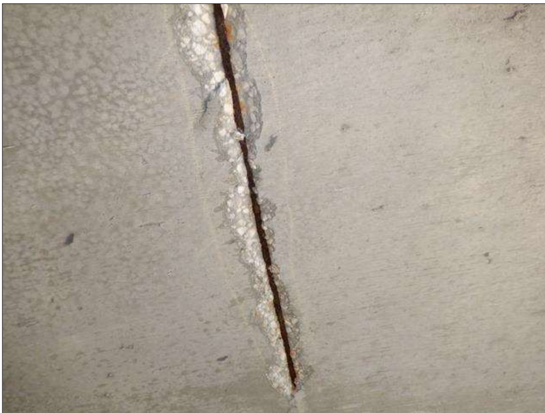
Span 5 Deck: 30" X 4" X 1" DEEP SPALL LOCATED ON BOTTOM SIDE OF DECK IN BAY 3 NEAR ENDBENT 2. EXPOSED REBAR
