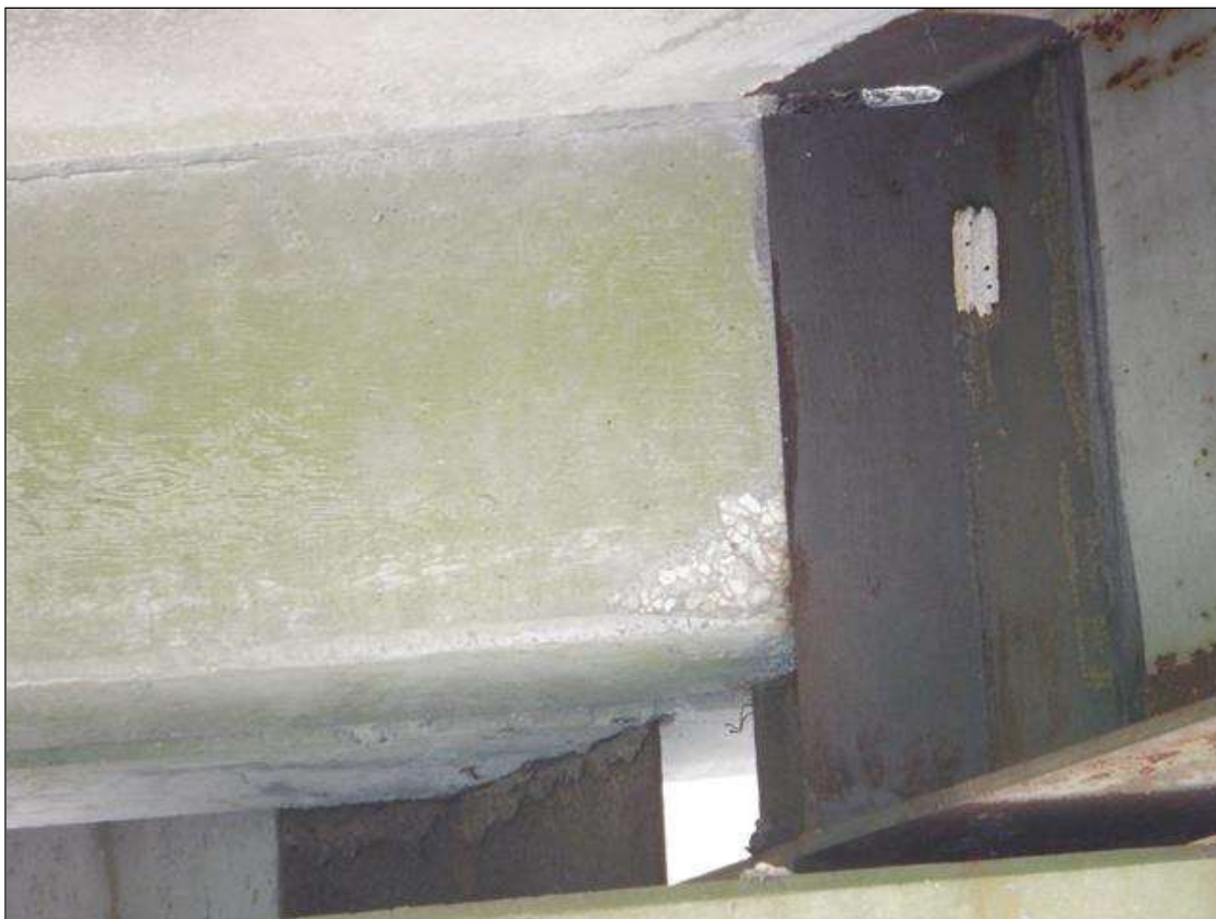
SPALL MEASURING 8" IN DIAMETER BY 1" DEEP LOCATED IN THE CONCRETE BUILD UP IN SPAN 1 BAY 2 OVER BENT 1.
