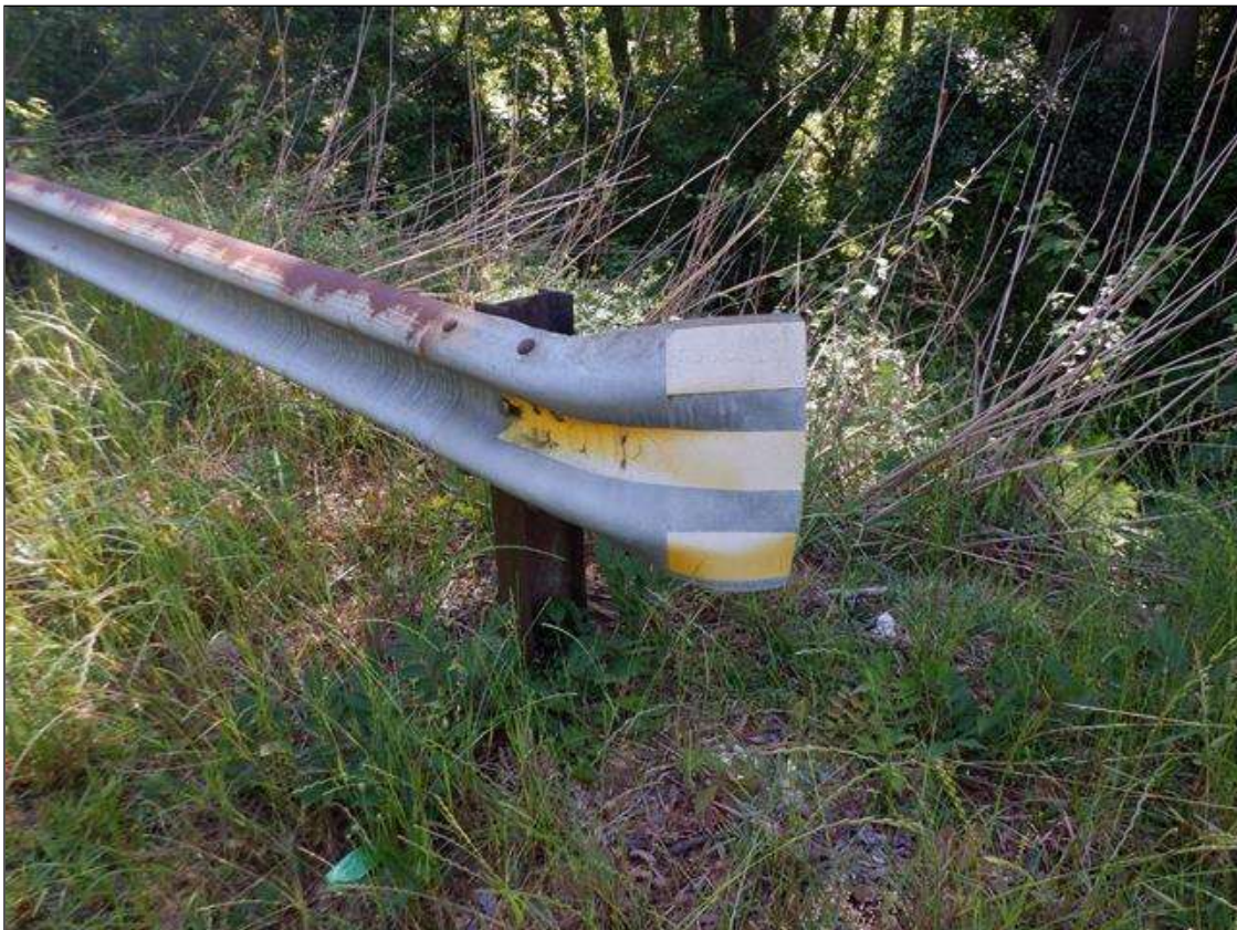
SW GUARDRAIL END TERMINAL
