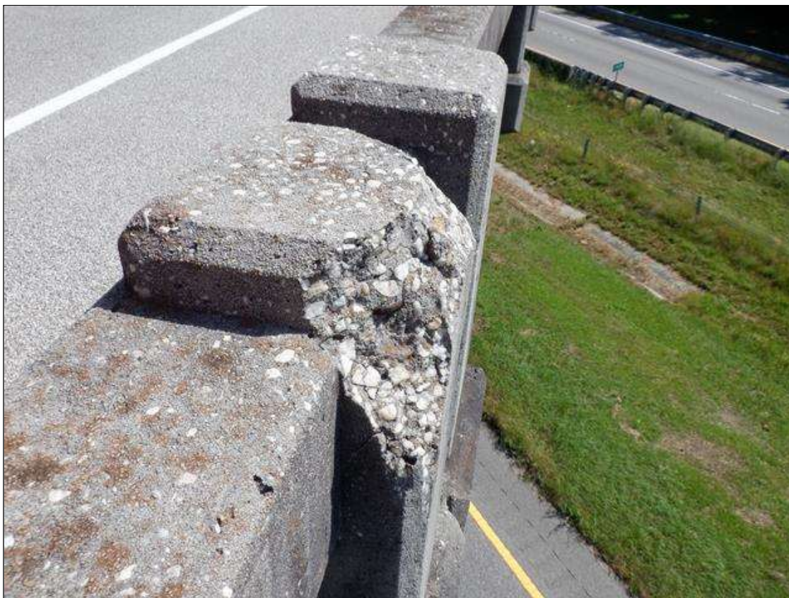
Span 2 Right Bridge Rail: RAIL POST # 4 SPALL 4" HIGH X 2" WIDE X 1" DEEP WITH EXPOSED REBAR
