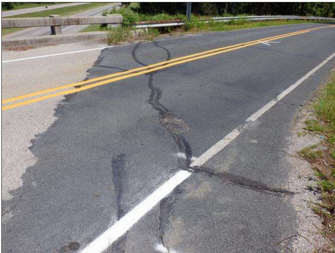
LAERAL CRACKING ACROSS ENTIRE ROADWAY 5FT EAST OF EAST APPROACH
