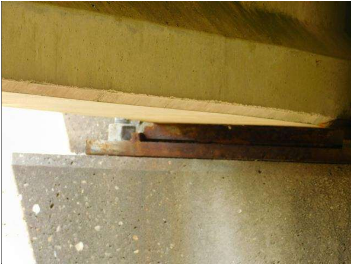
Span 5 Beam 4 Near Bearing: SURFACE CORROSION
