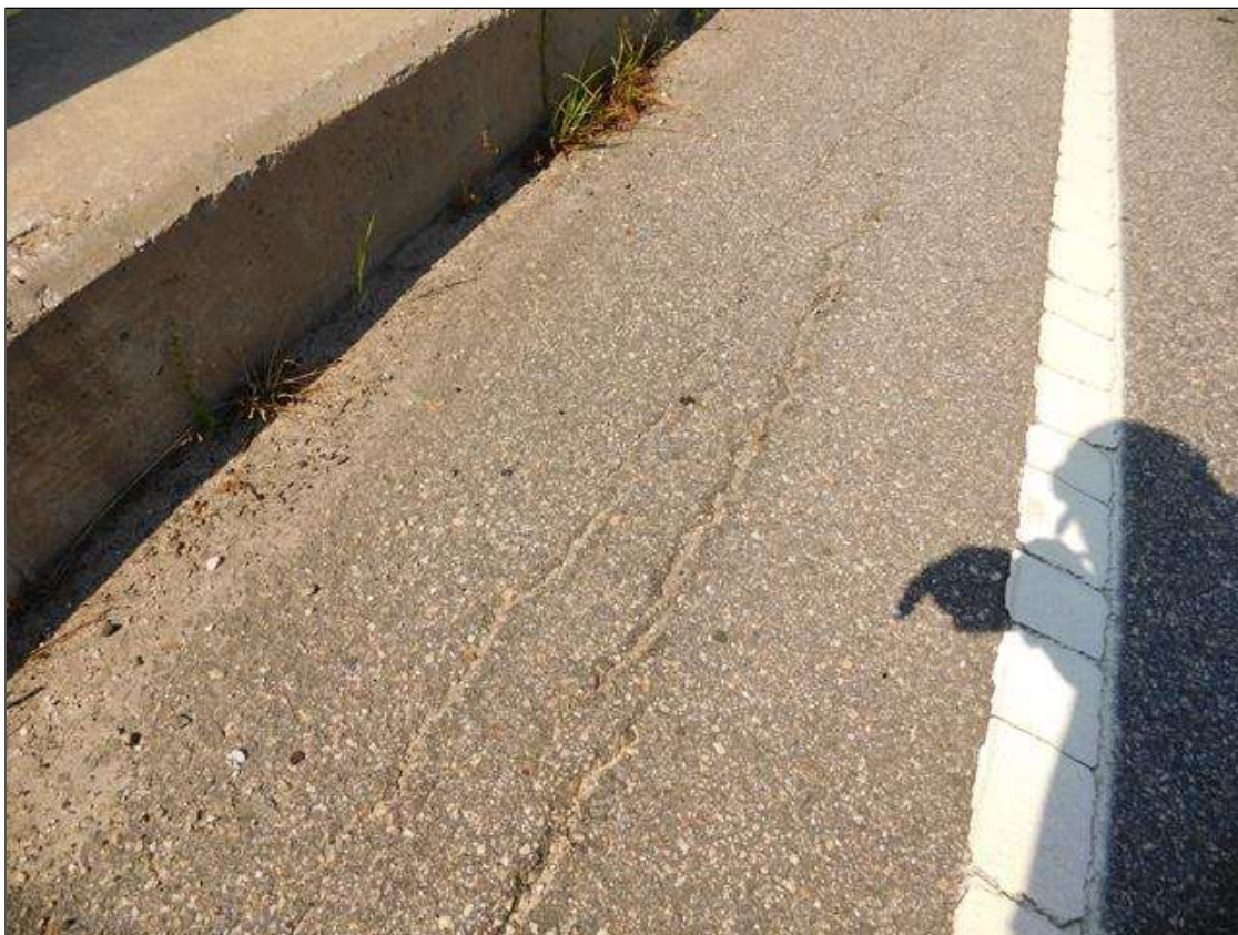
Span 2 Wearing Surface: 50 FT. LONGITUDINAL CRACK .005 WIDE IN RIGHT SHOULDER
