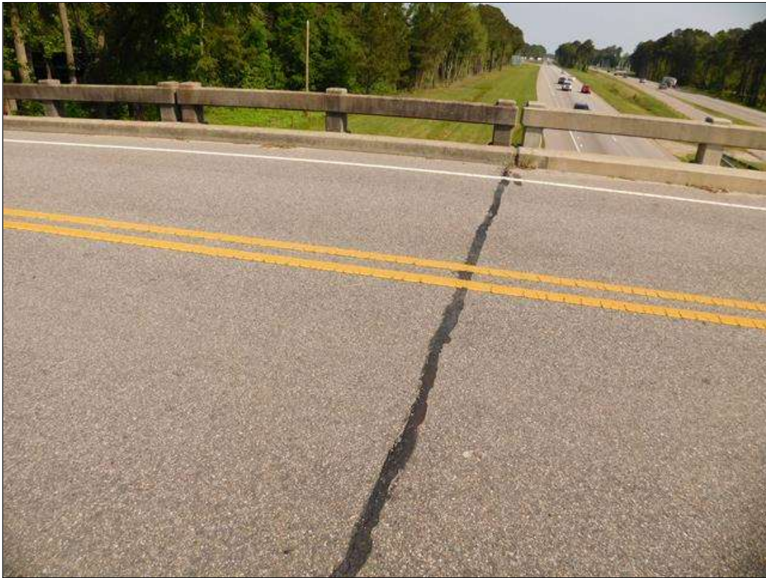
Span 2 Wearing Surface: 24 FT. SEALED TRANSVERSE CRACK OVER BENT 1
