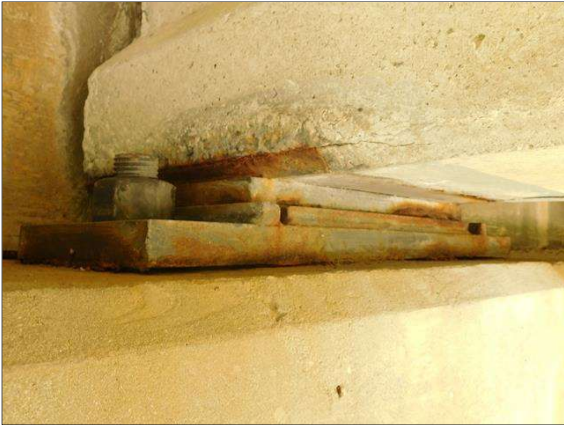
Span 3 Beam 3 Near Bearing: SURFACE CORROSION
