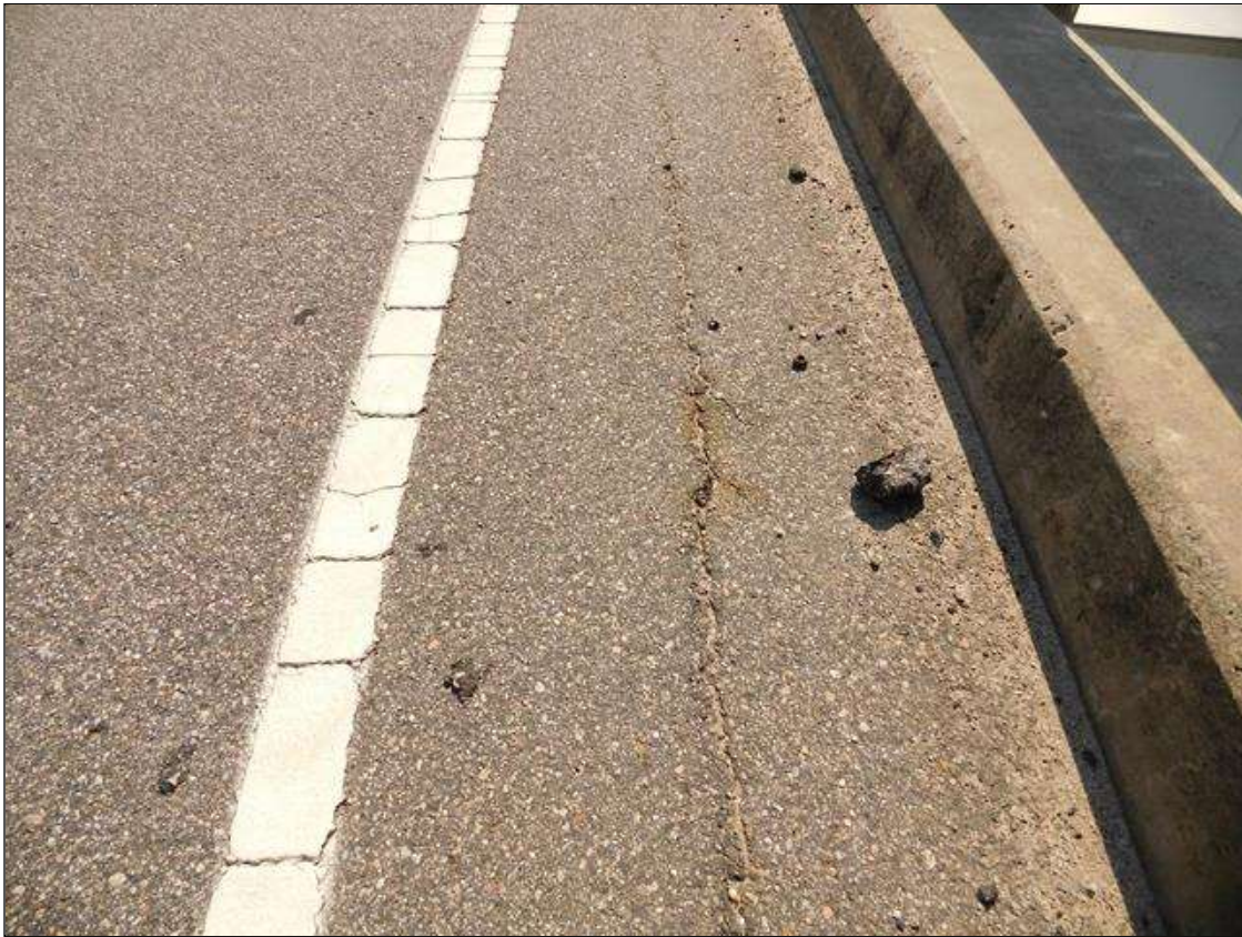
Span 4 Wearing Surface: .010 LONGITUDINAL CRACK IN THE RIGHT SHOULDER
