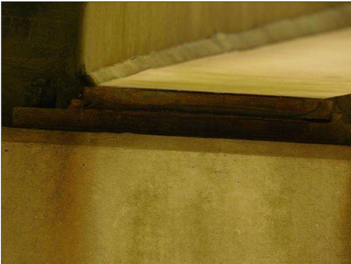
Span 1 Beam 3 Far Bearing: RUST AND FLAKING WITH NO SECTION LOSS
