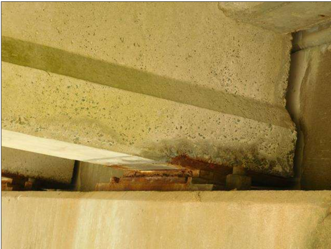
Span 3 Beam 2 Near Bearing: RUST AND FLAKING WITH NO SECTION LOSS
