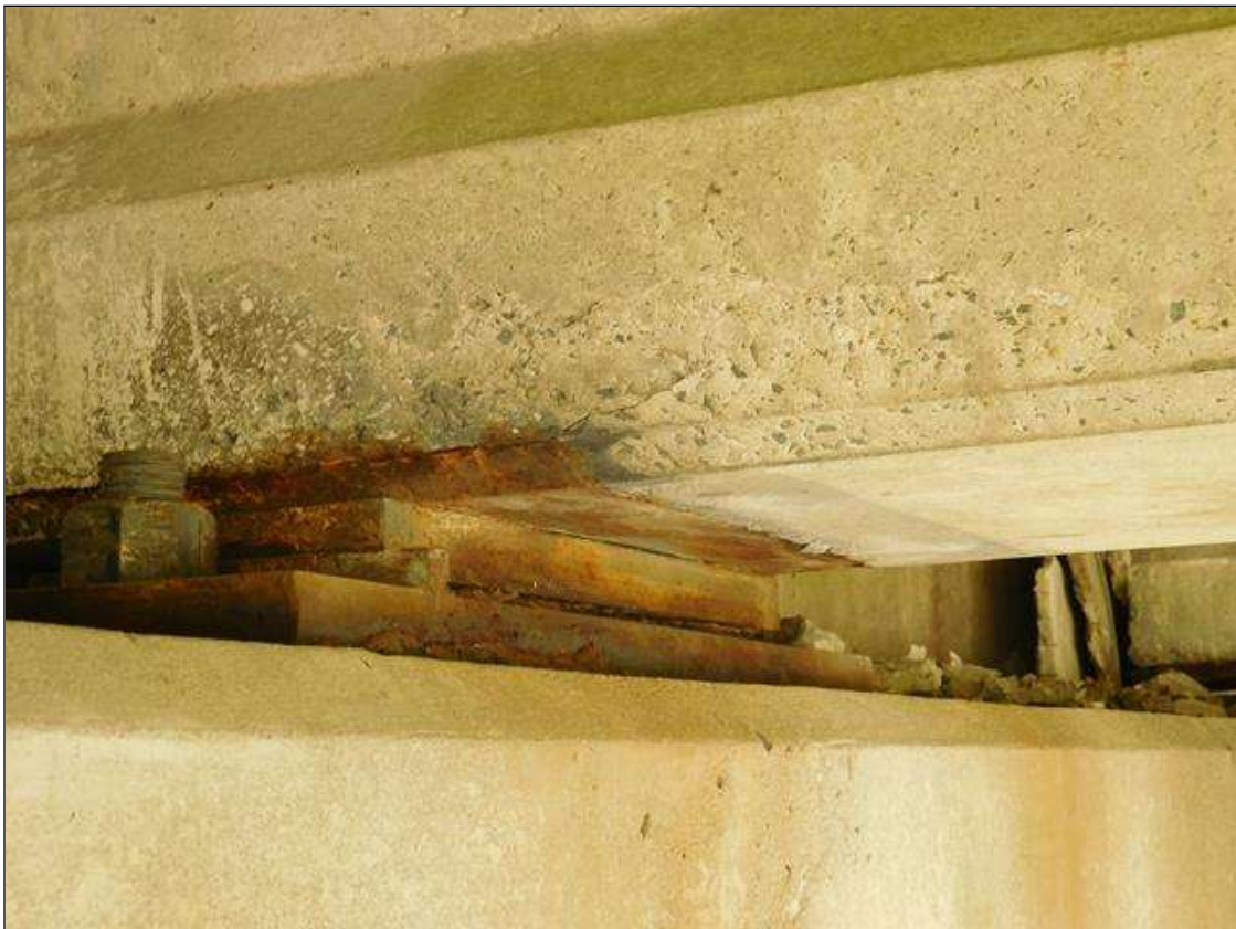
Span 3 Beam 2 Far Bearing: RUST AND FLAKING WITH NO SECTION LOSS
