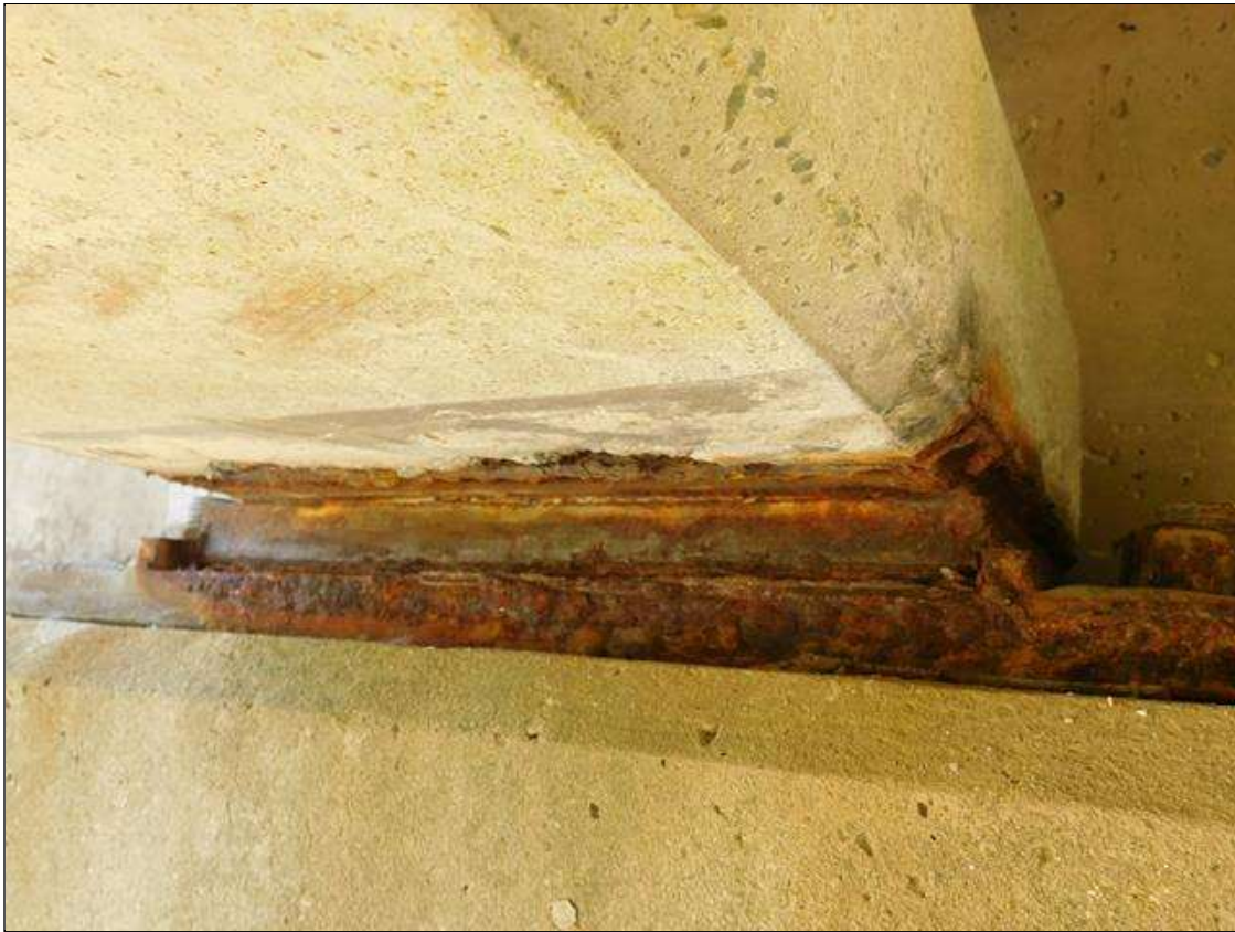
Span 3 Beam 1 Far Bearing: 1/8" OF PACK RUST
