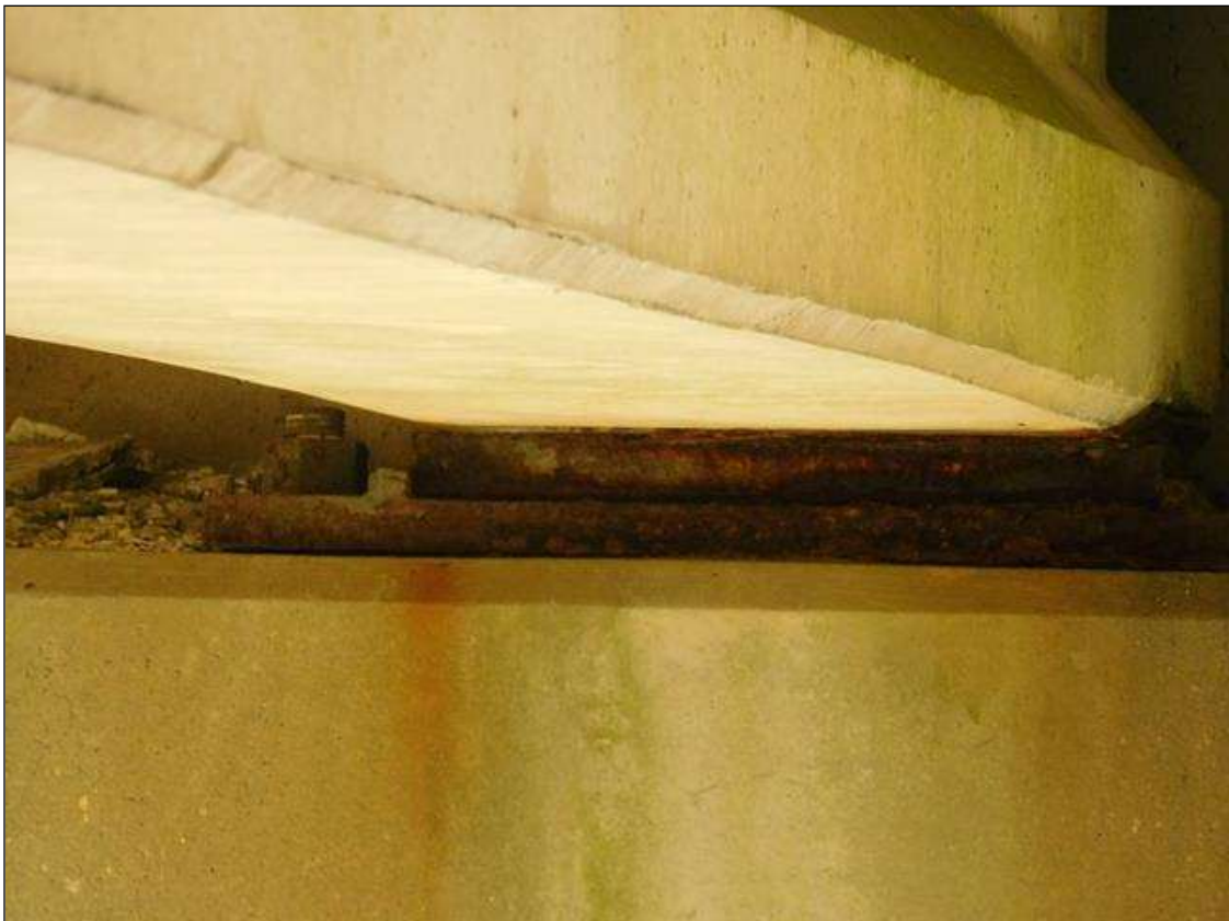
Span 5 Beam 3 Near Bearing: RUST AND FLAKING WITH NO SECTION LOSS
