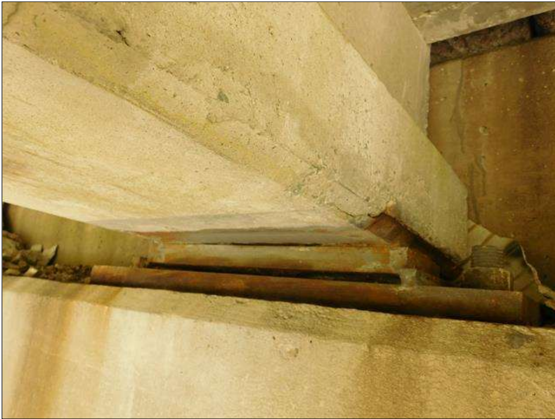
Span 3 Beam 3 Far Bearing: SURFACE CORROSION
