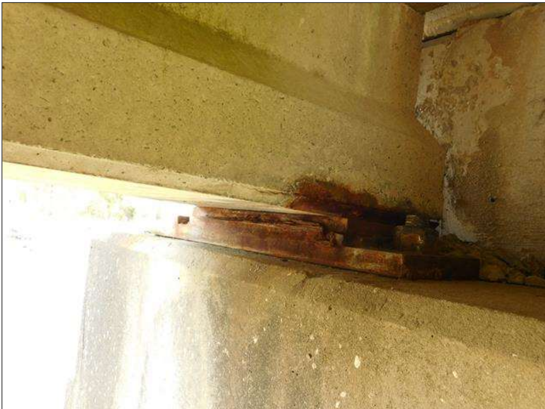
Span 3 Beam 4 Near Bearing: RUST AND FLAKING WITH NO SECTION LOSS
