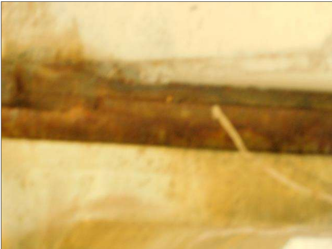
Span 5 Beam 4 Far Bearing: RUST AND FLAKING WITH NO SECTION LOSS
