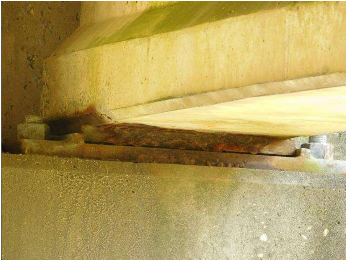
Span 5 Beam 1 Near Bearing: RUST AND FLAKING WITH NO SECTION LOSS
