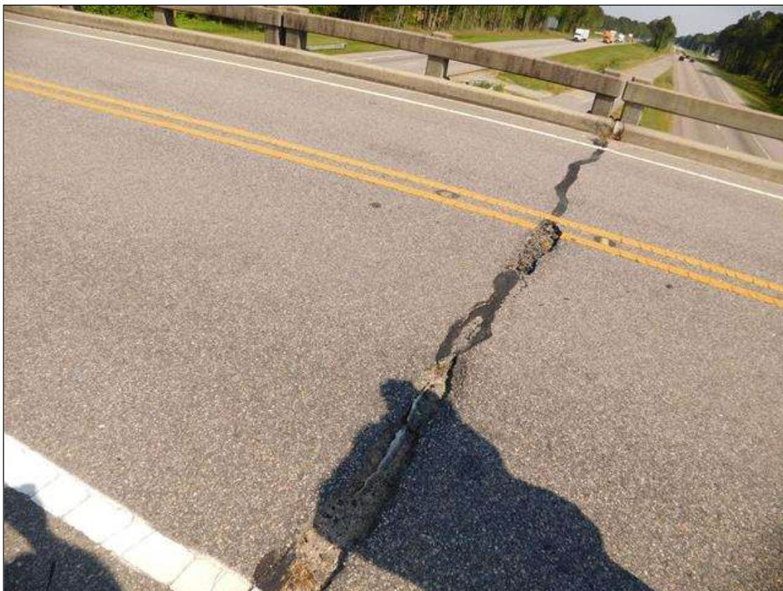
Span 4 Wearing Surface: 2 - 36" WIDE X UP TO 8" LONG X 2" DEEP POTHOLES AT BENT 3 IN THE EASTBOUND LANE
