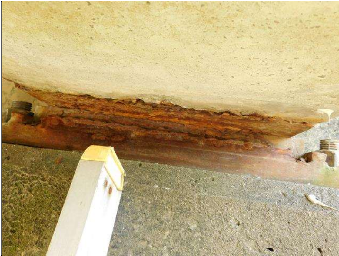
Span 3 Beam 1 Near Bearing: 1/8" OF PACK RUST
