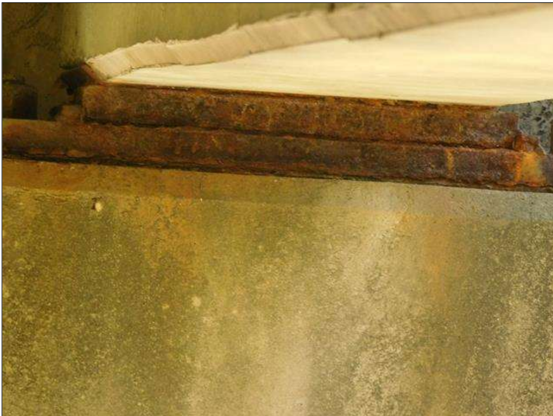
Span 1 Beam 4 Far Bearing: RUST AND FLAKING WITH NO SECTION LOSS
