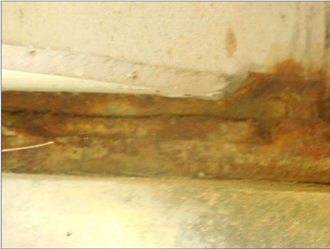
Span 1 Beam 4 Near Bearing: RUST AND FLAKING WITH NO SECTION LOSS
