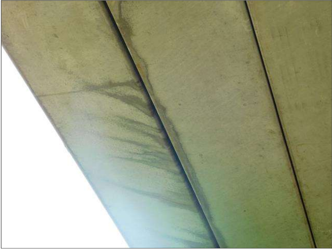
Span 2 Slab 1: 50 FT. OF EFFLORESCENCE LEAKAGE BETWEEN UNITS 1 AND 2
