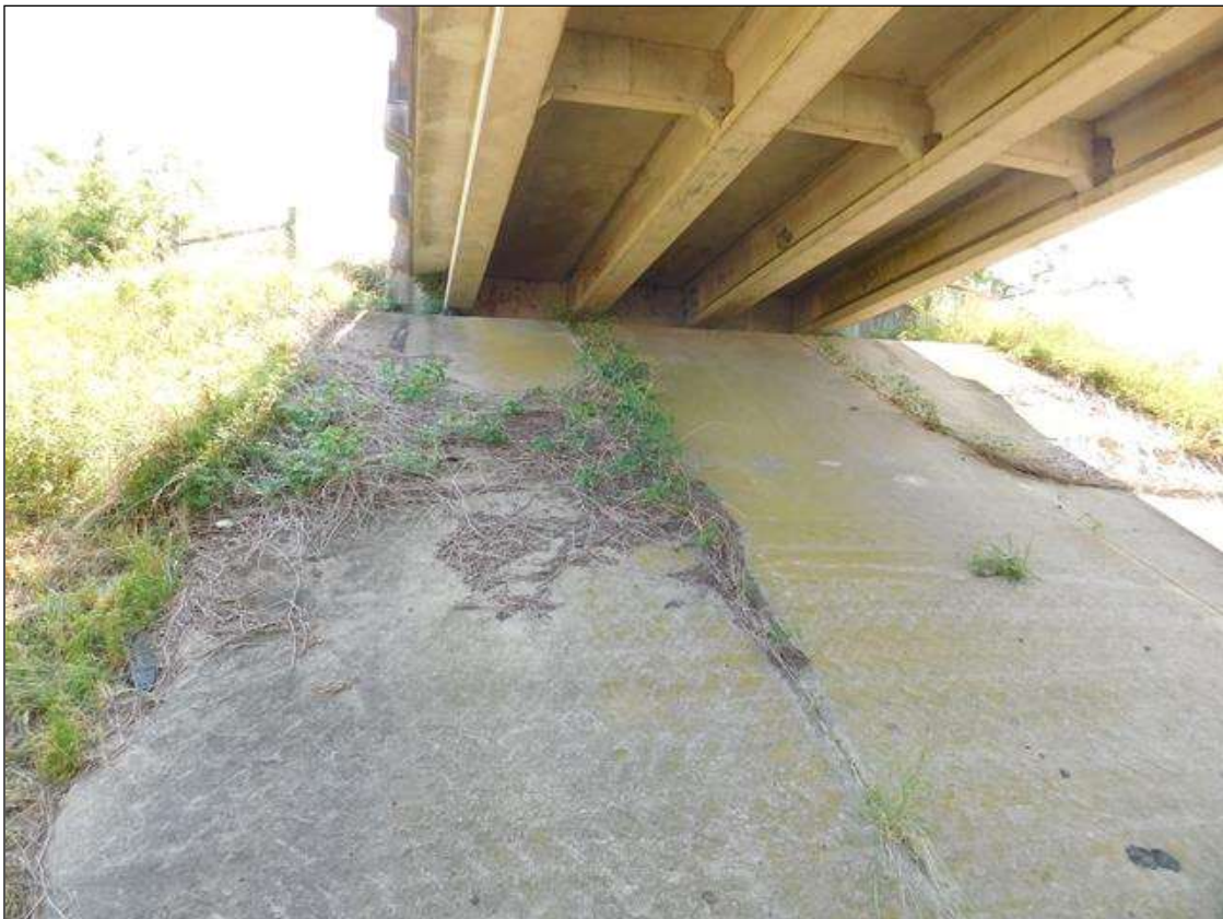
VEGETATION ON END BENT 2 SLOPE, 75 SQUARE FOOT. FT.
