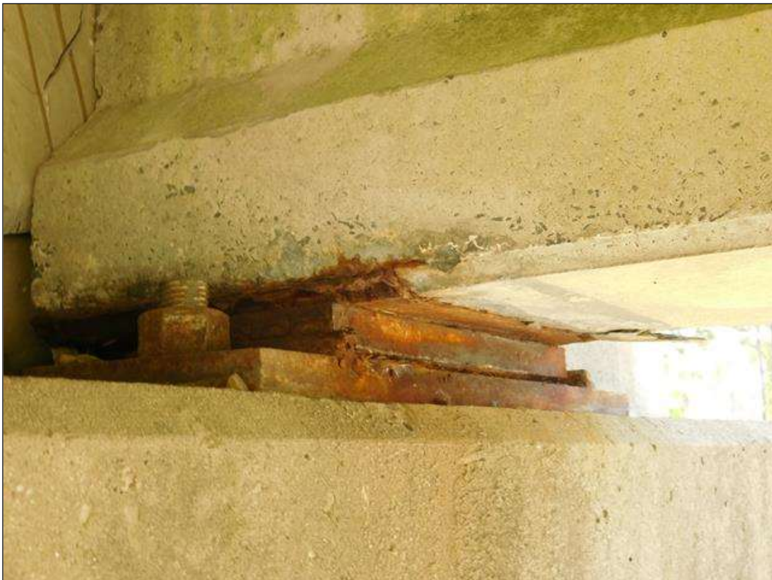
Span 3 Beam 4 Far Bearing: RUST AND FLAKING WITH NO SECTION LOSS
