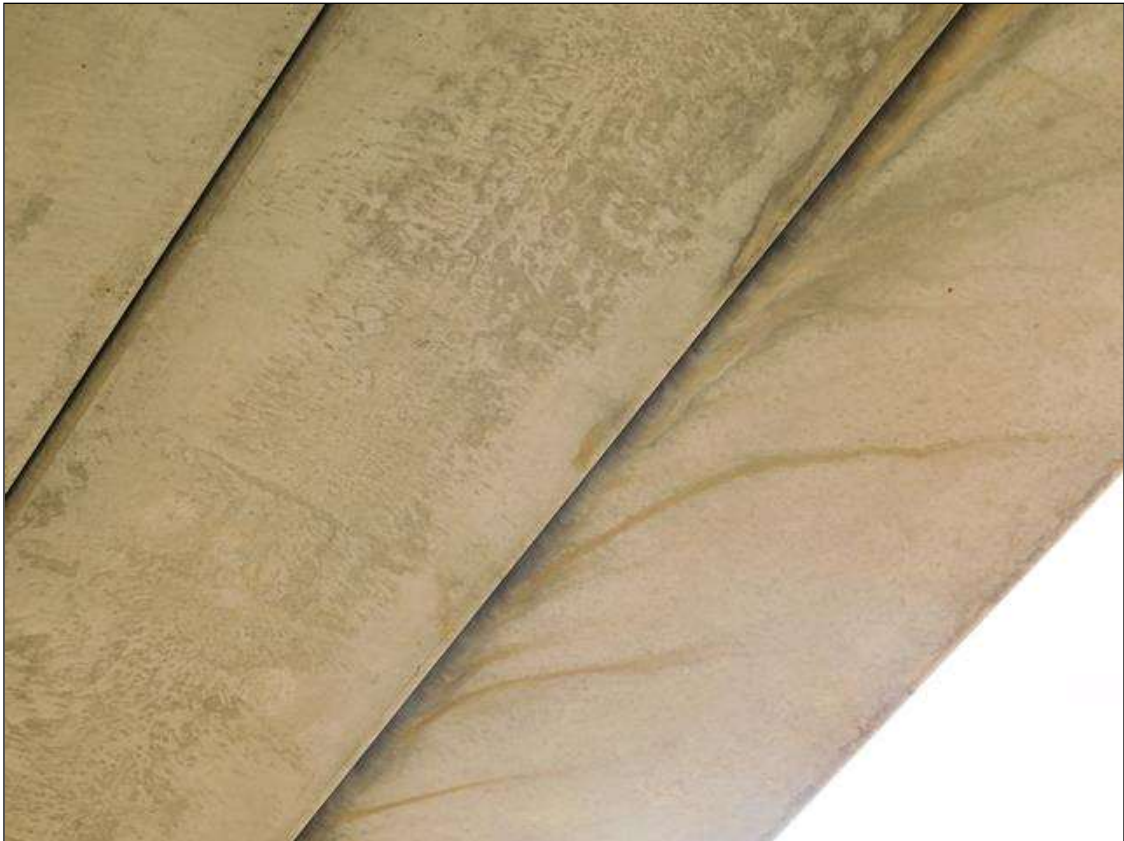
Span 2 Slab 8: 50 FT. OF EFFLORESCENCE LEAKAGE BETWEEN UNITS 8 AND 9
