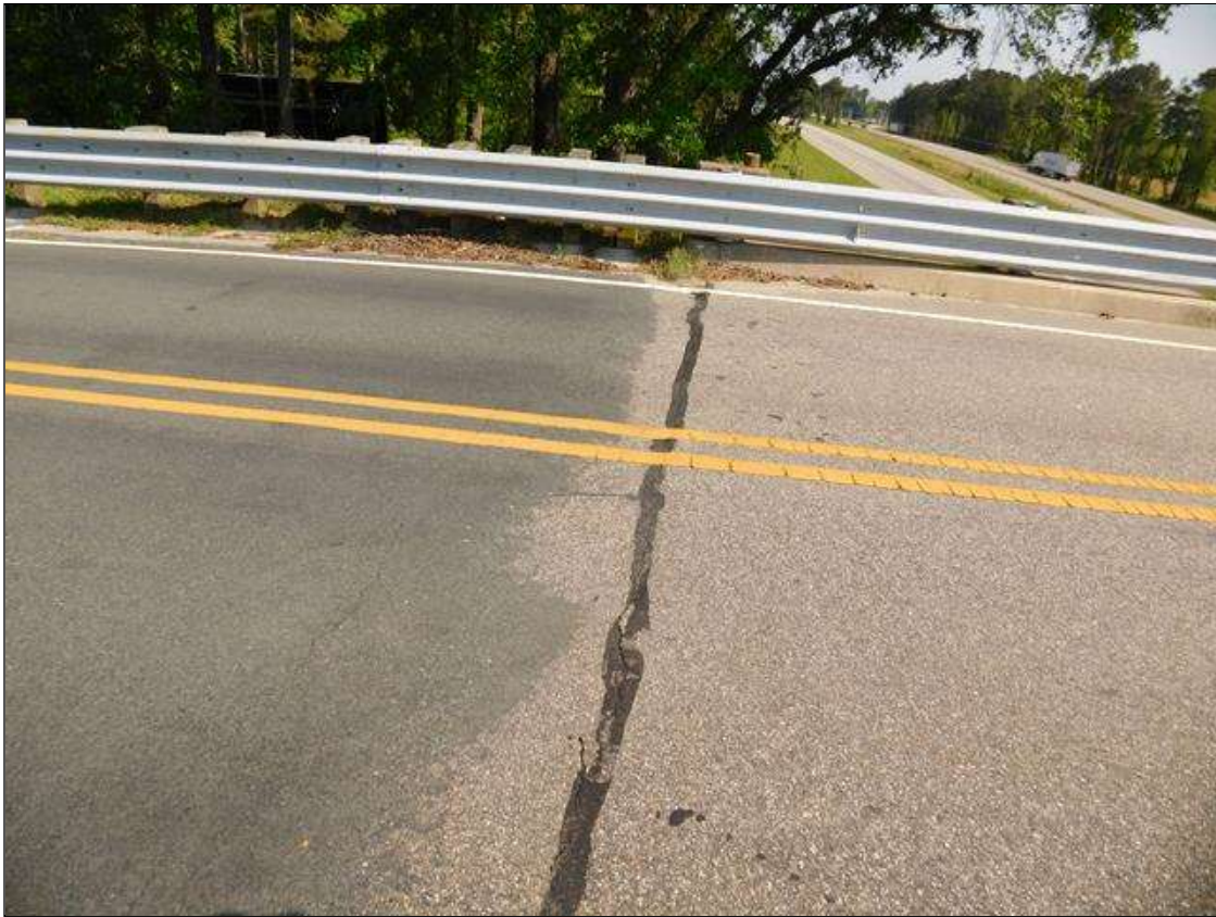
Span 1 Wearing Surface: 24 FT. LONG SEALED CRACK AT END BENT 1
