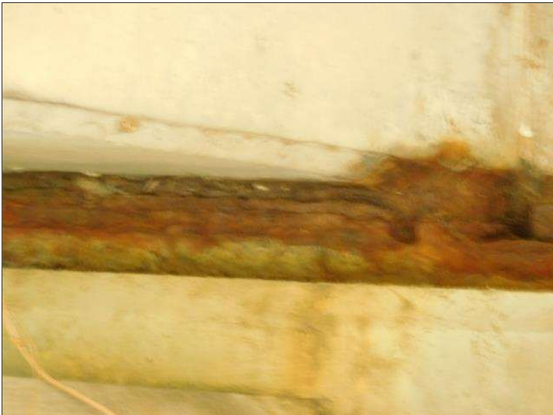
Span 5 Beam 1 Far Bearing: 1/8" OF PACK RUST
