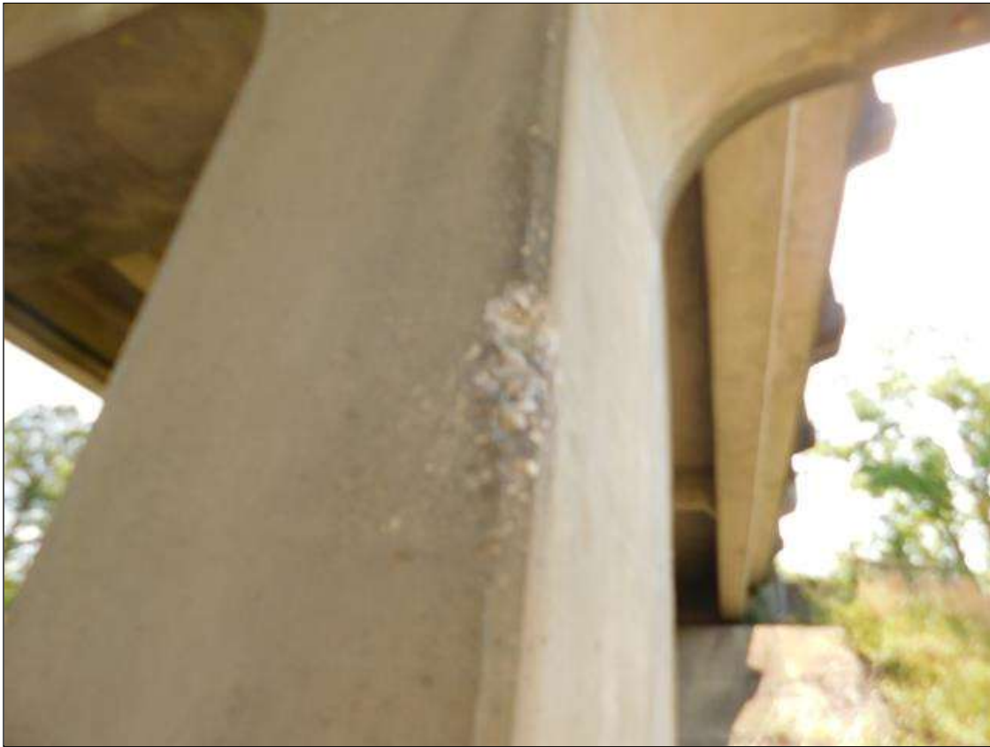
Bent 4 Pile 2: SPALL 8" HIGH X 2" WIDE X 2" DEEP AT EAST FACE 5 FT. BELOW CAP
