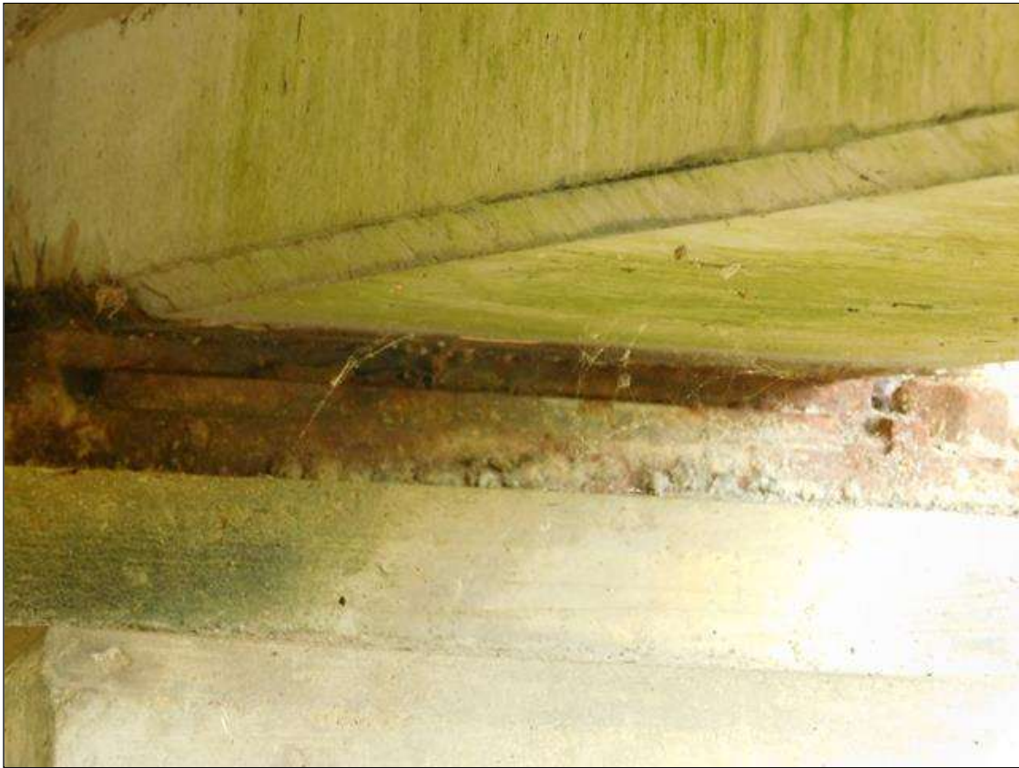
Span 1 Beam 1 Near Bearing: RUST AND FLAKING WITH NO SECTION LOSS
