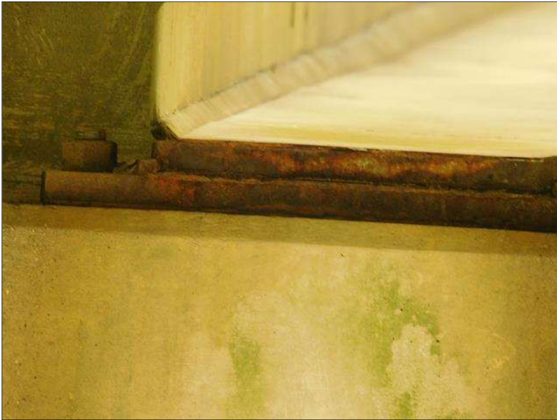
Span 1 Beam 2 Far Bearing: RUST AND FLAKING WITH NO SECTION LOSS
