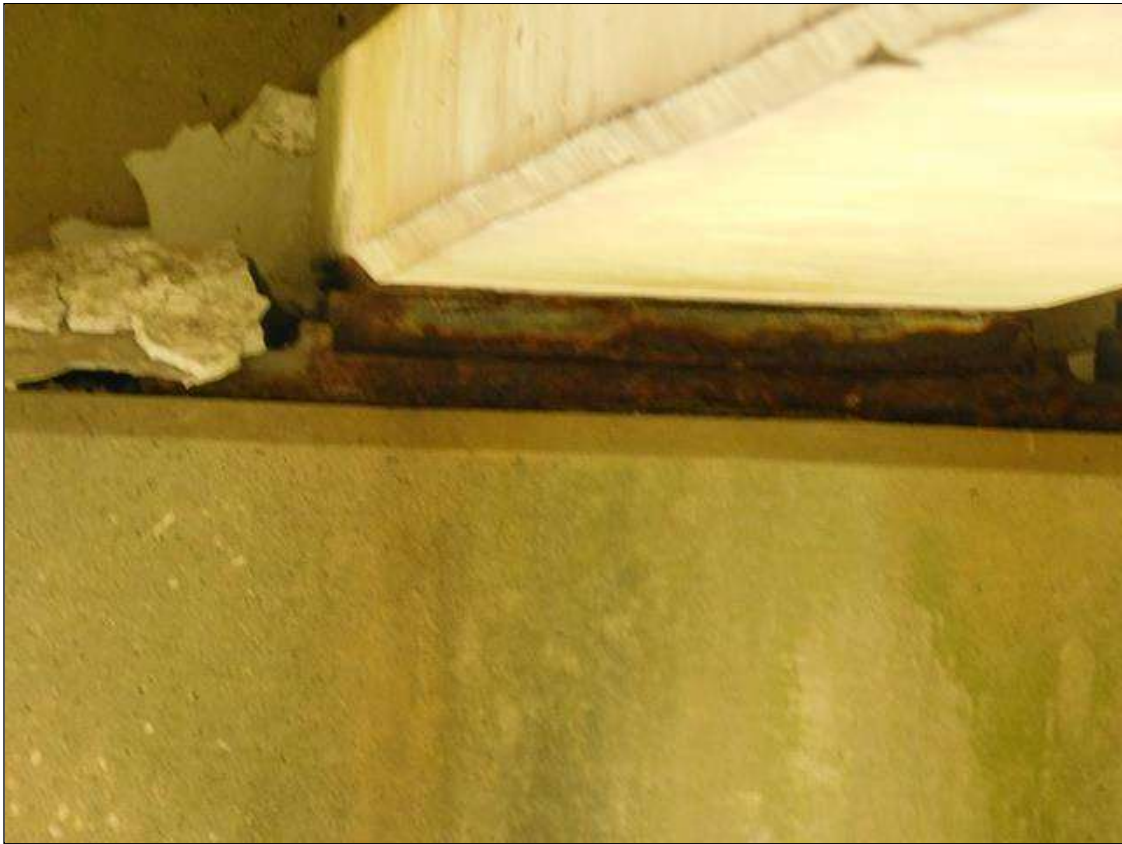
Span 5 Beam 2 Near Bearing: RUST AND FLAKING WITH NO SECTION LOSS
