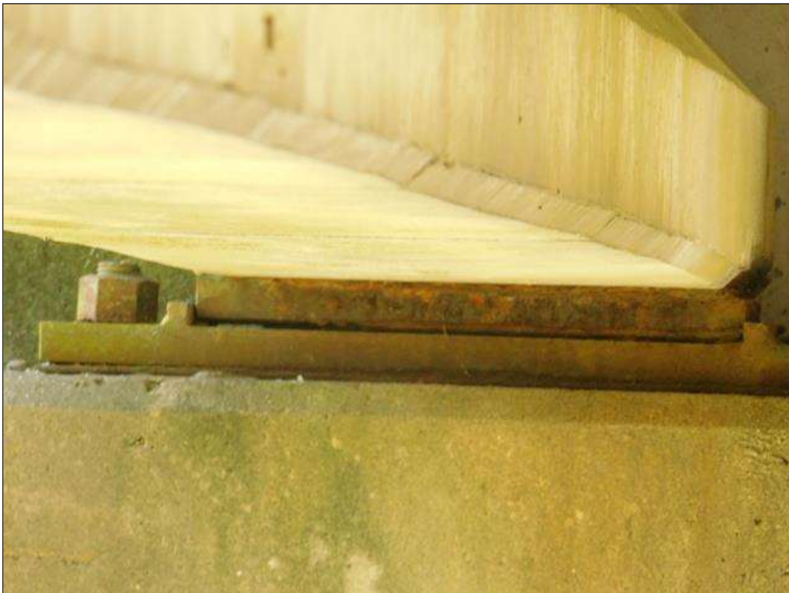
Span 1 Beam 1 Far Bearing: RUST AND FLAKING WITH NO SECTION LOSS
