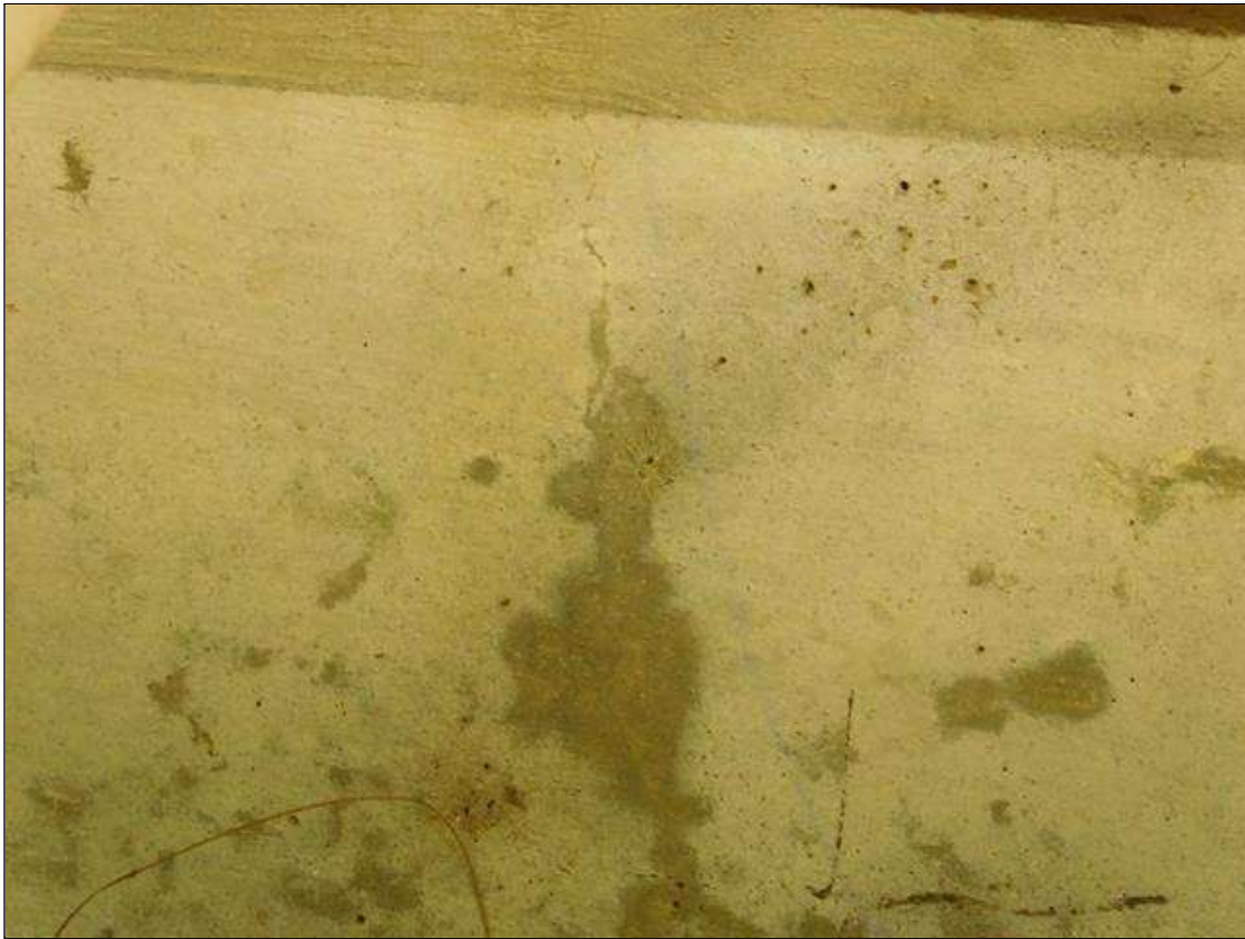
End Bent 1 Cap 1: 12" VERTICAL HAIRLINE CRACK UNDER BAY 1
