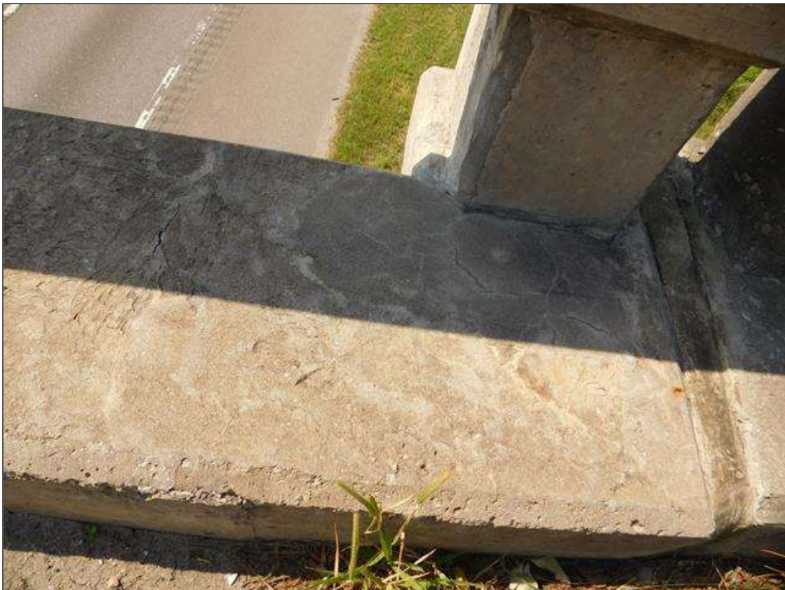
Span 2 Right Bridge Rail: 2 SF. OF HAIRLINE MAP CRACKING IN TOP OF CURB AT BENT 1
