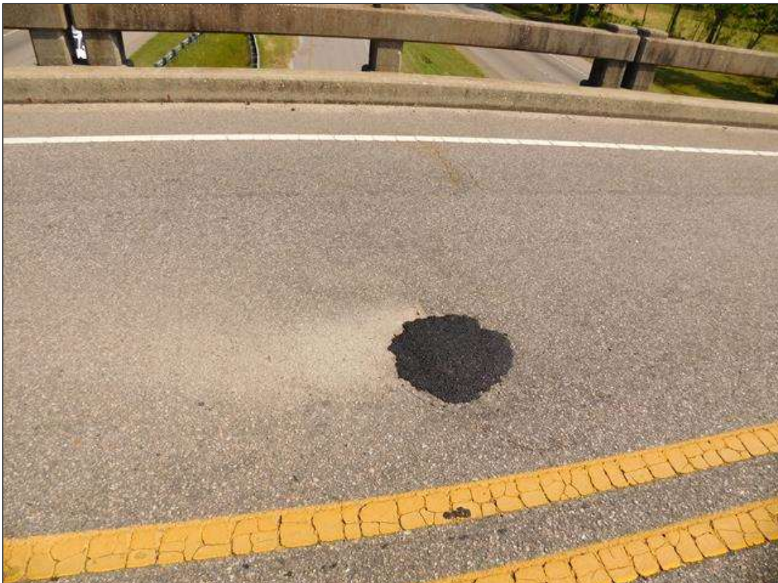
Span 3 Wearing Surface: SOUND PATCH IN WESTBOUND LANE AT MIDSPAN
