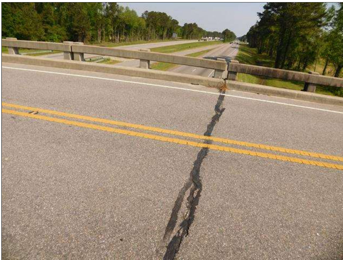
Span 5 Wearing Surface: SEALED TRANSVERSE CRACK OVER BENT 4
