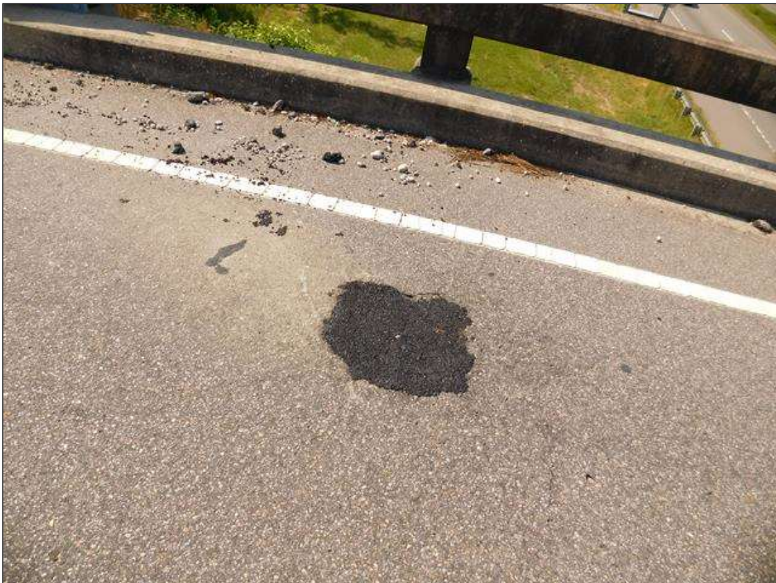
Span 5 Wearing Surface: 1 FT. PATCH IN EASTBOUND LANE AT MID SPAN
