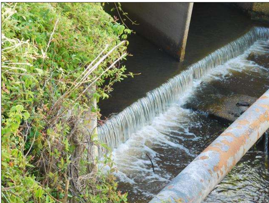
Barrel 2 Section 1: SCOUR AT WEST OUTLET END 10 FT. WIDE X 1 FT. DEEP WITH NO UNDERMINING
