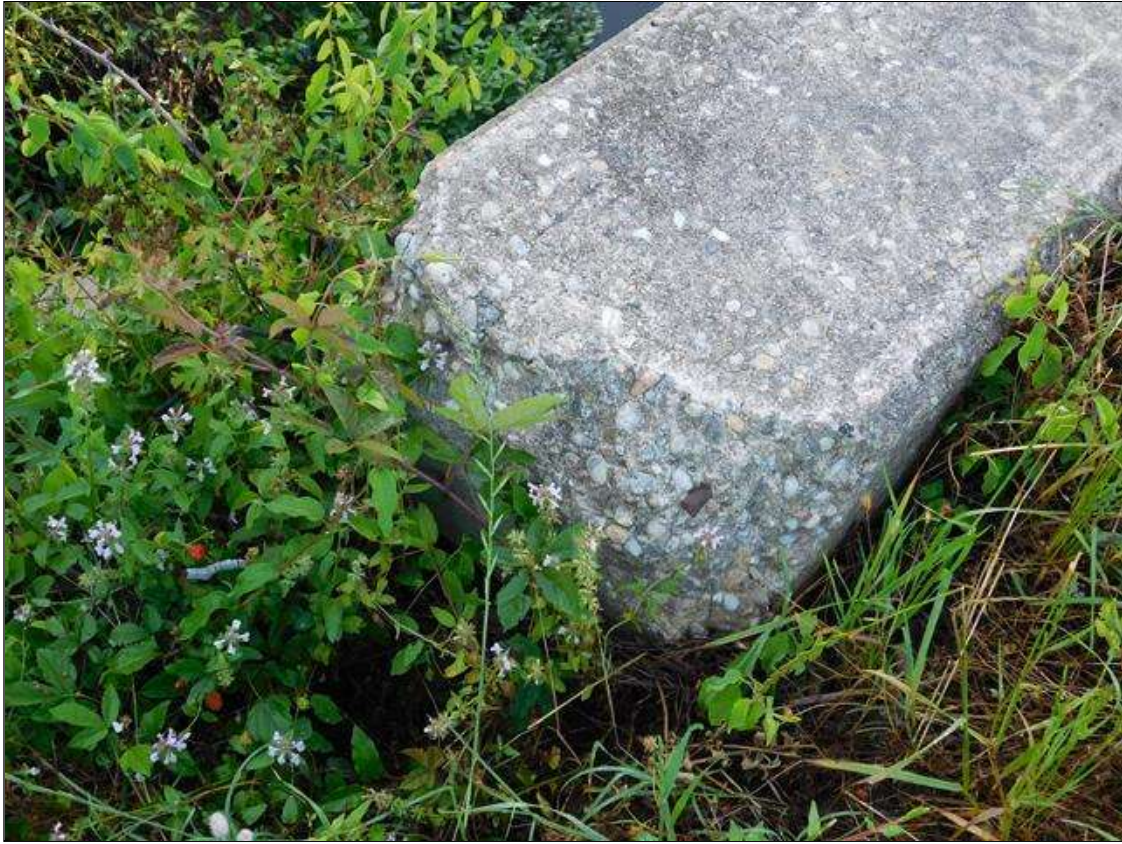
NORTHEAST CORNER , EAST HEADWALL SPALLED 18" WIDE X 5" HIGH X UP TO 4" DEEP
