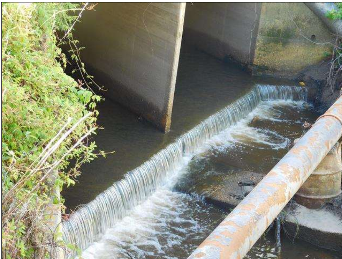
Barrel 1 Section 1: SCOUR AT WEST OUTLET END 10 FT. WIDE X 1 FT. DEEP WITH NO UNDERMINING
