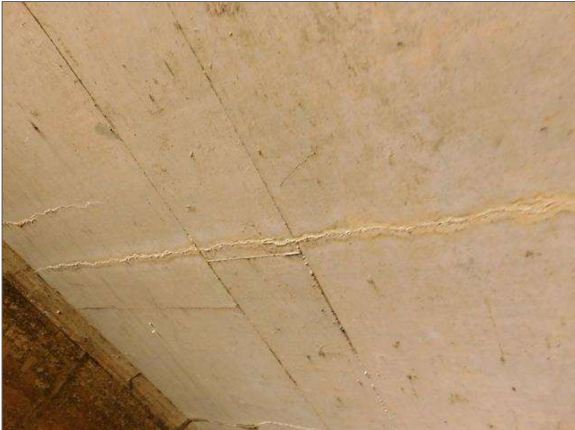
Barrel 2 Section 1: HAIRLINE LONGITUDINAL CRACKS WITH EFFLO IN TOP SLAB 10' SPACING STARTING AT 30' FROM EAST END
