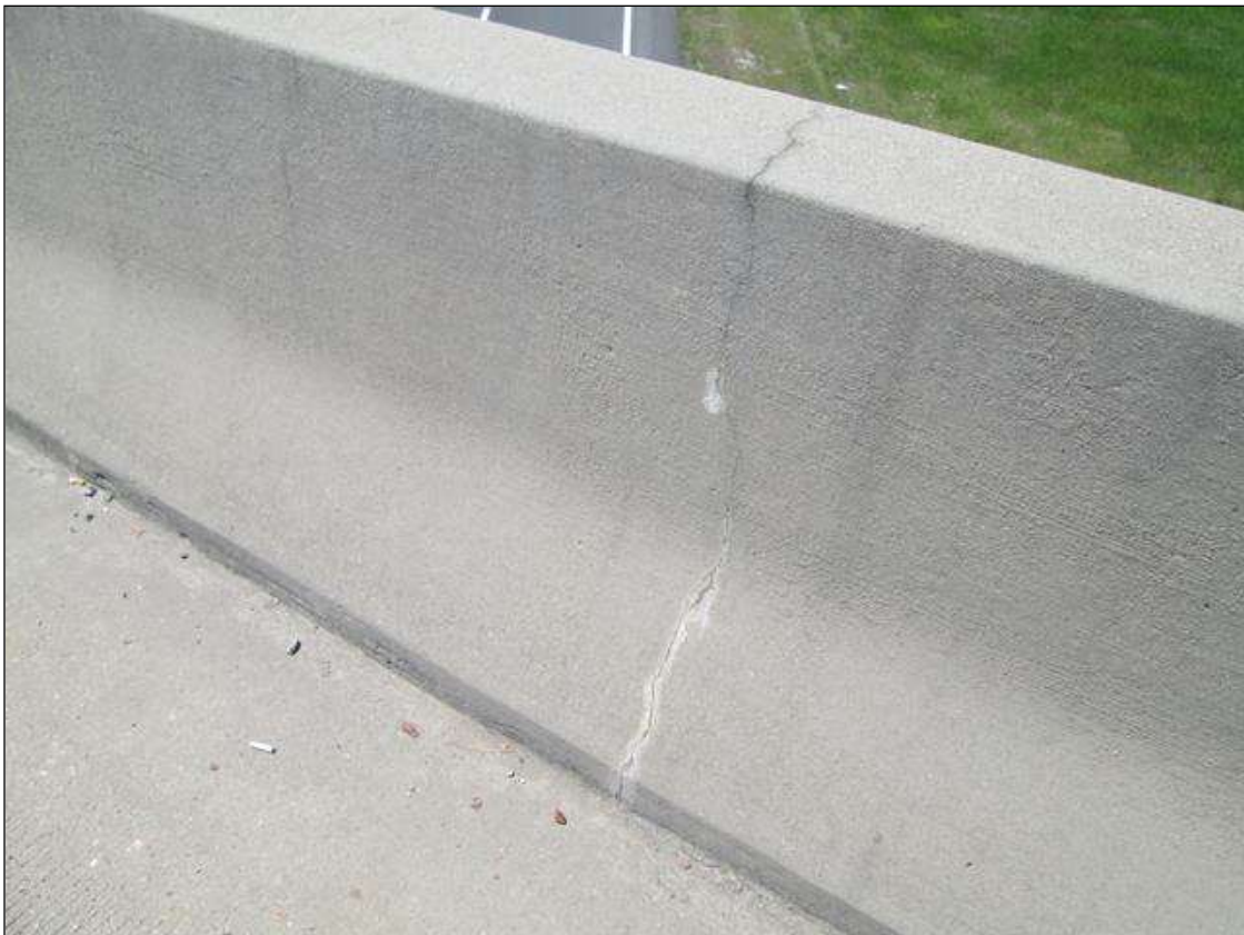
Span 2 Right Bridge Rail: SCATTERED VERTICAL CRACKS WITH EFFLO STAINS.
