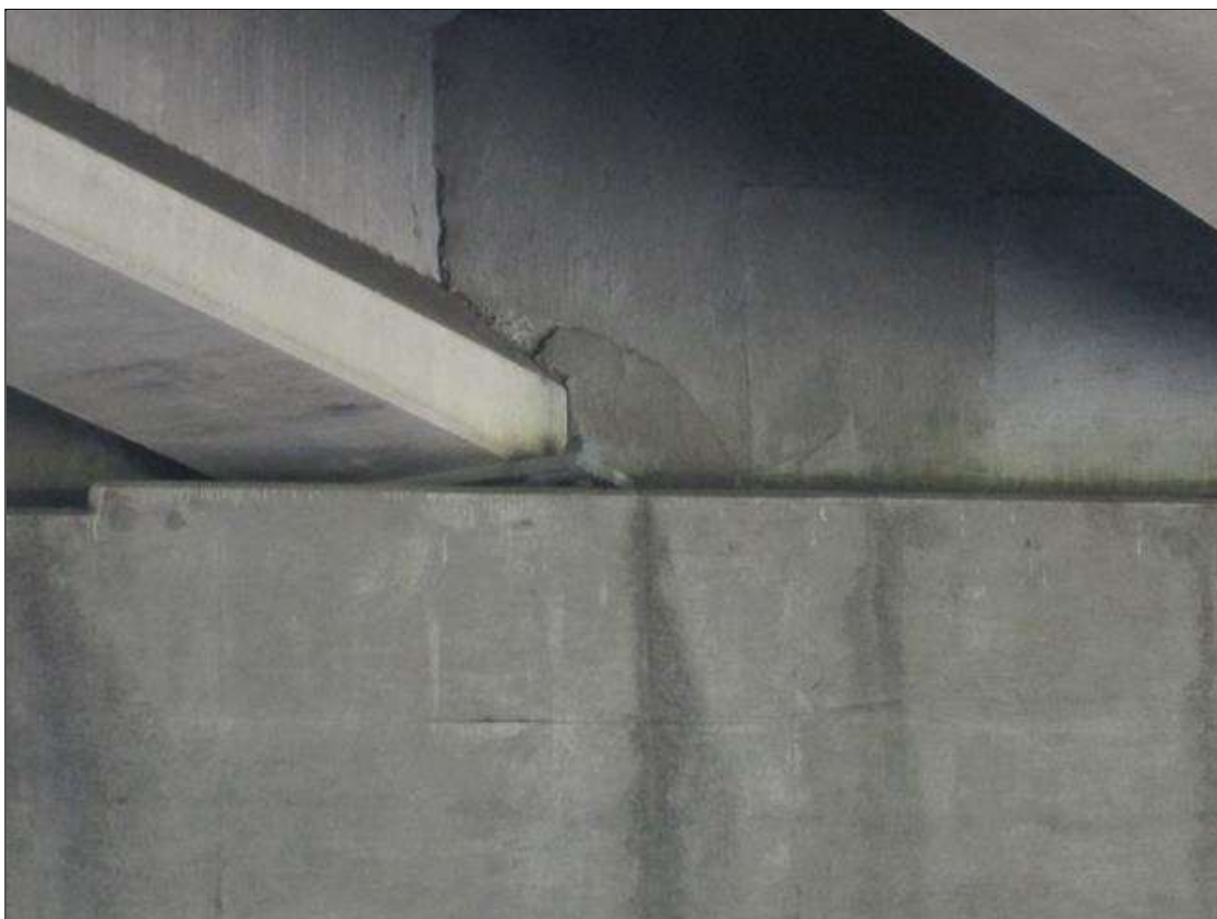
END DIAPHRAGM IN SPAN 3 OVER BENT 2 EAST FACE AT LT SIDE G7 HAS DELAMINATED AREA 12" X 16".
