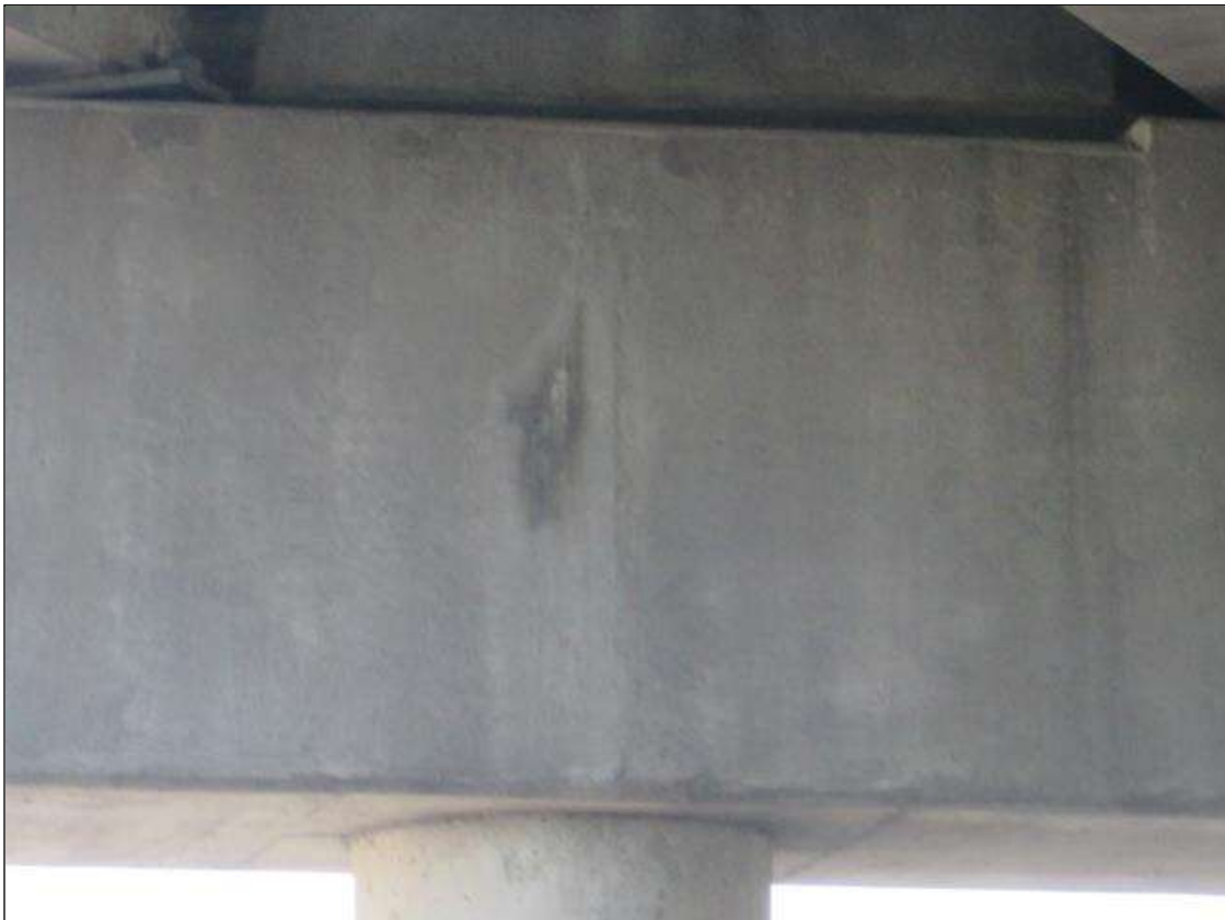
Bent 2 Cap 1: BENT 2 EAST FACE OF CAP HAS VERTICAL CRACK WITH EFFLO STAIN BETWEEN G11 AND G12.
