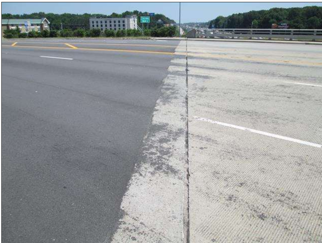
Expansion Joint : DIRT AND SMALL GRAVEL INSIDE JOINT OVER END BENT 1.
