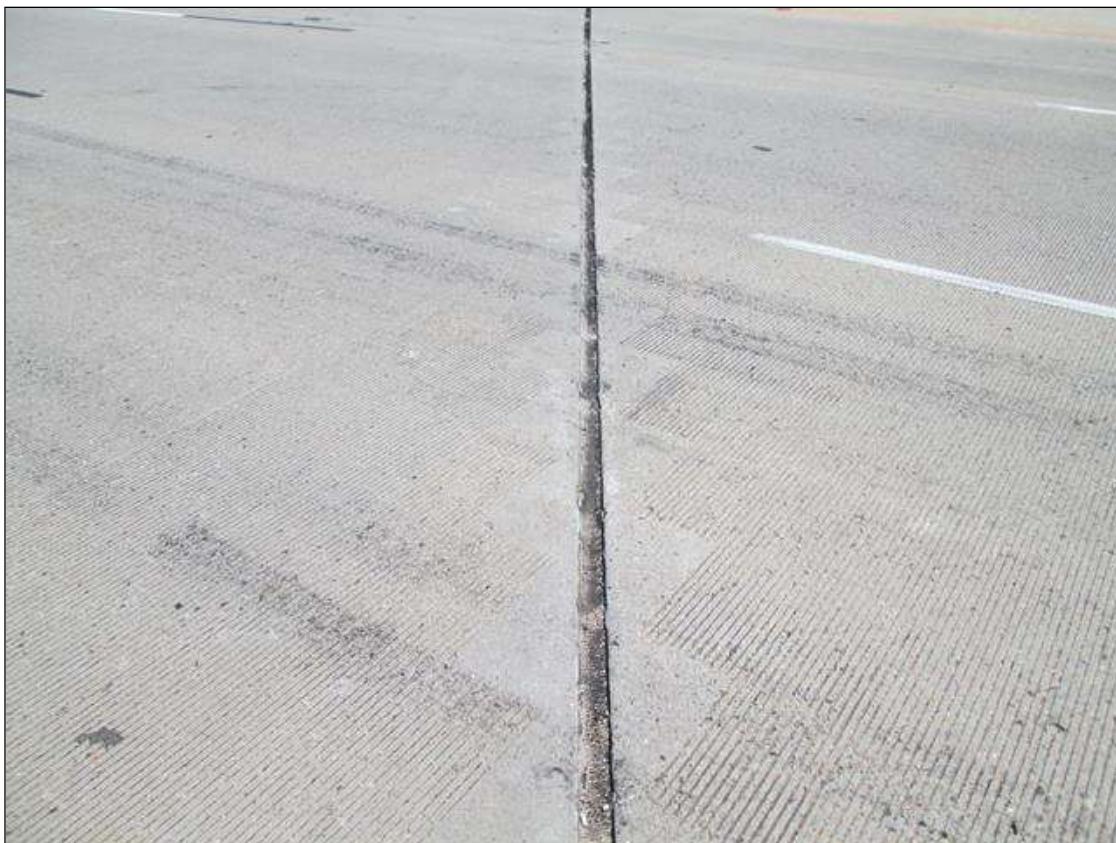
Expansion Joint : DIRT AND SMALL GRAVEL INSIDE THE JOINT OVER BENT 3.
