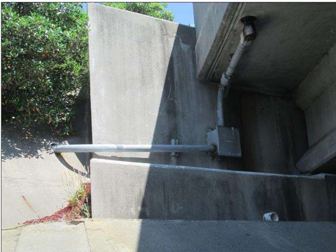
UTILITY IS ATTACHED AT THE RT ABUT OUTSIDE G12 AT END BENT 1 AND END BENT 2 SIMILAR AREA.
