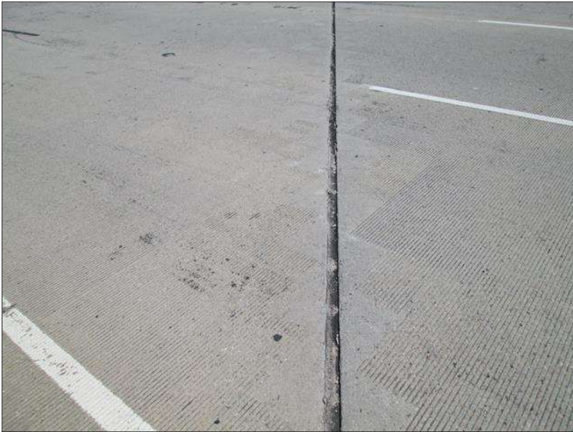
Expansion Joint : DIRT AND SMALL GRAVEL INSIDE JOINT.
