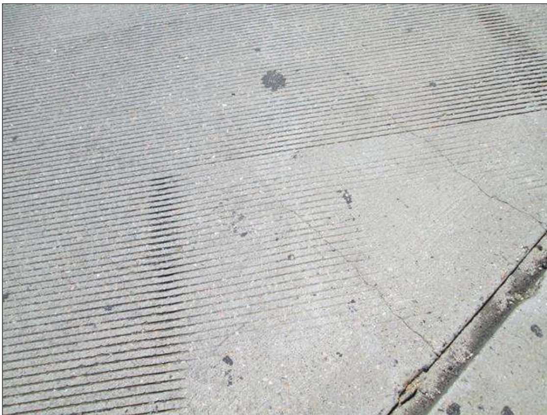
Span 1 Deck: SCATTERED LONGITUDINAL CRACKS AND SOME MAP CRACKING EXTENDING FROM END BENT 2 JOINT .
