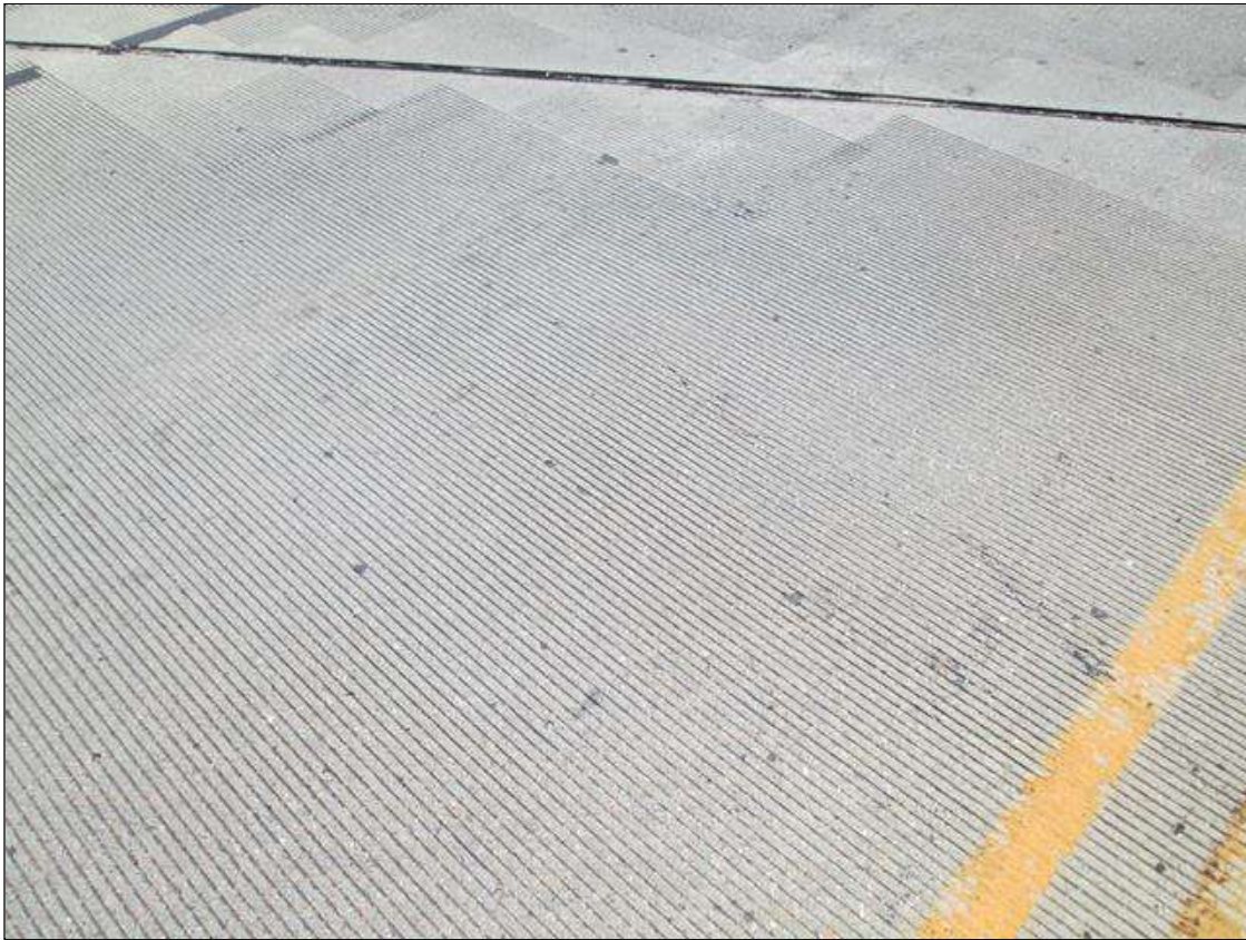
Span 1 Deck: TOP DECK IN SPAN 1 HAS SOME MAP CRACKING AND DIAGONAL CRACKS IN WBL COMING FROM JOINT AT BENT 1.
