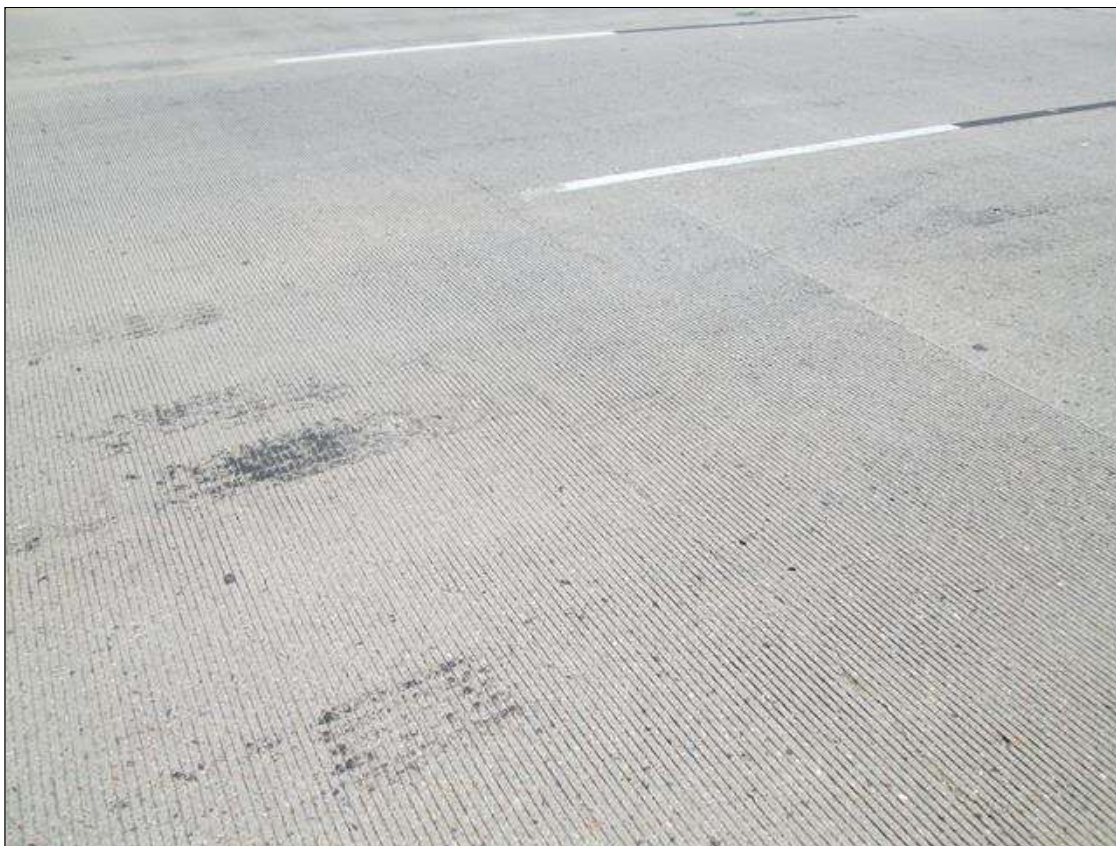
Span 3 Deck: SCATTERED TRANSVERSE CRACKS FROM 2' TO 5' CENTERS THROUGH OUT EBLs.
