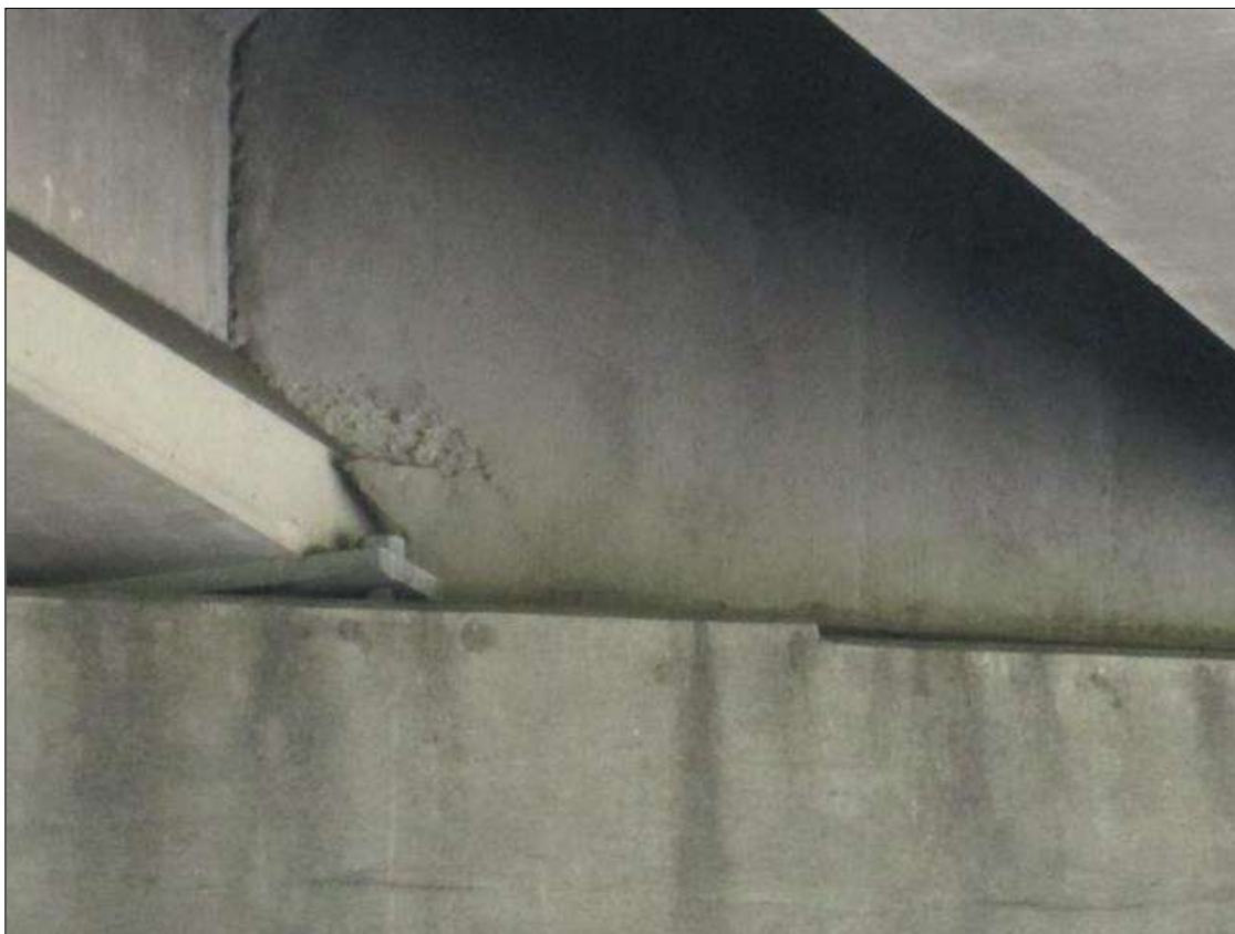
END DIAPHRAGM IN SPAN 3 OVER BENT 2 EAST FACE IN BAY 5 AT LT SIDE OF G6 HAS DELAMINATED AND SPALLED AREA 12" X 14".
