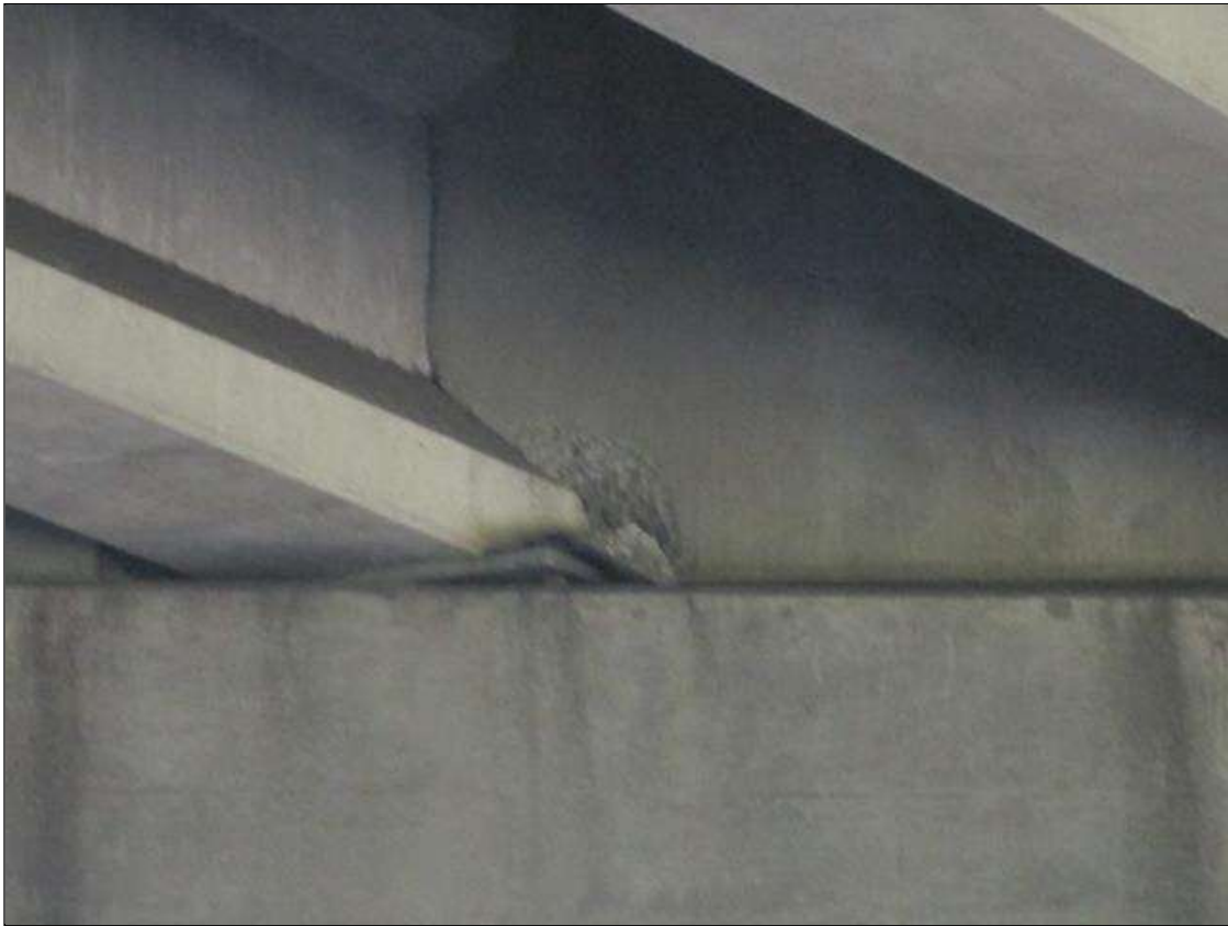
END DIAPHRAGM IN SPAN 3 OVER BENT 2 EAST FACE ON LT SIDE OF G8 HAS SPALLED AREA 8" X 12" X 2" DEEP.
