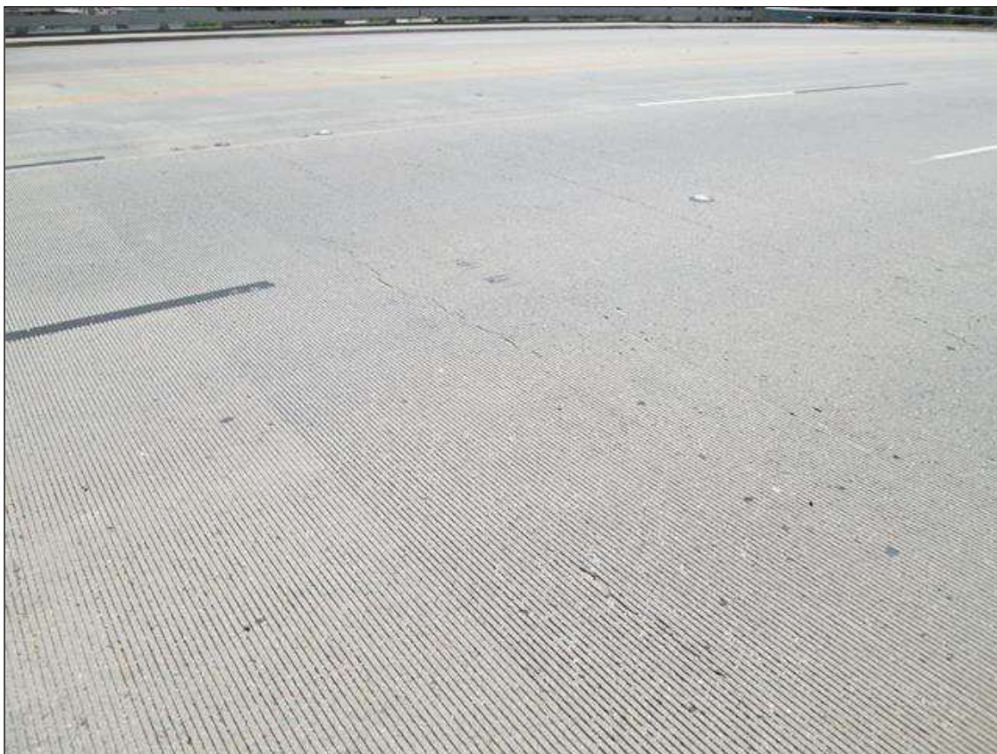
Span 2 Deck: TOP OF THE DECK IN SPAN 2 SOME MAP CRACKING AND TRANSVERSE CRACKS FROM 2' TO 5' ON CENTERS THROUGH OUT EBLs .
