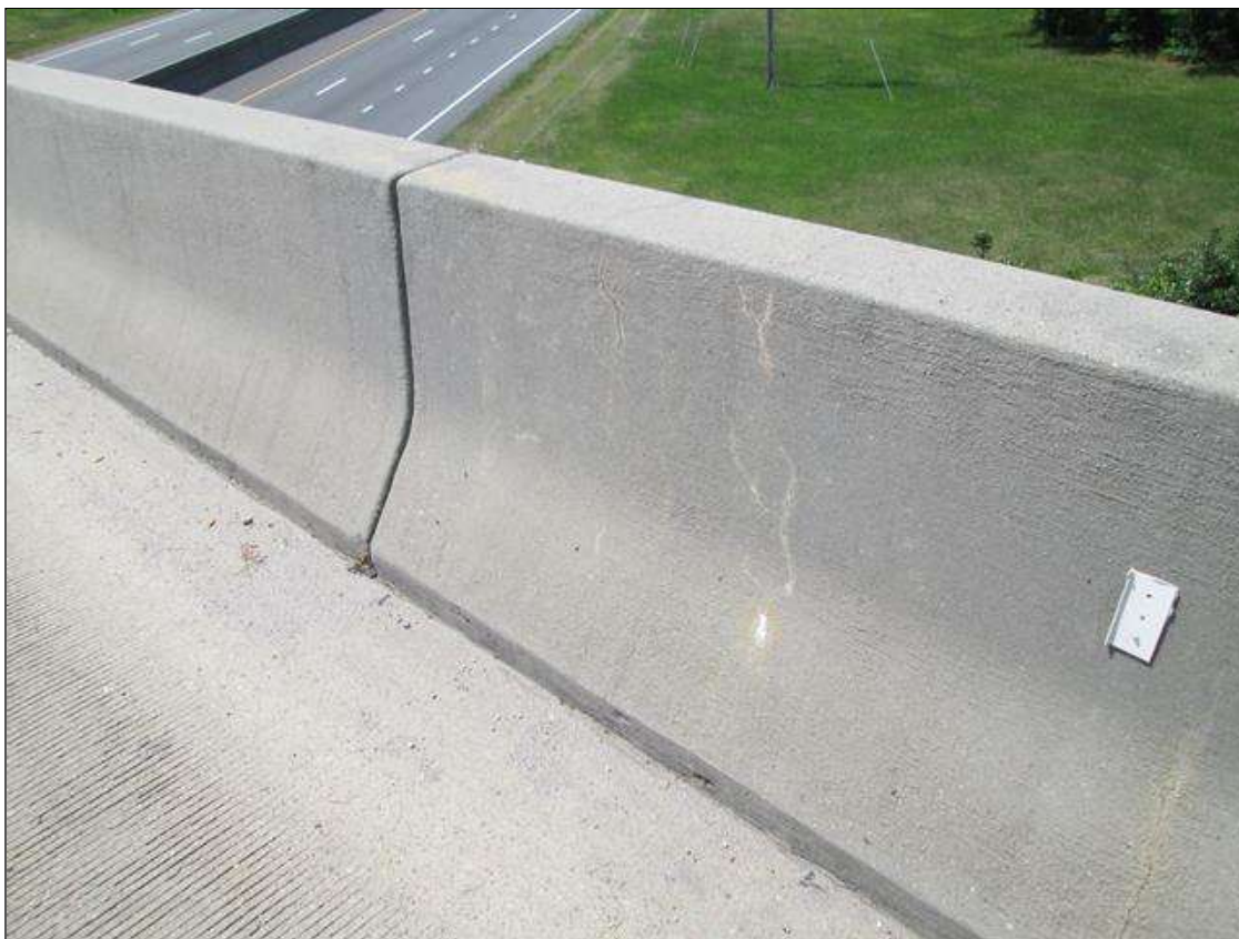
Span 1 Right Bridge Rail: SCATTERED VERTICAL CRACKS WITH EFFLO STAINS.
