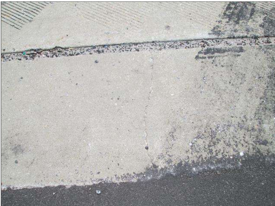
Approach 1: SCATTERED LONGITUDINAL CRACKS IN WEST APPROACH .
