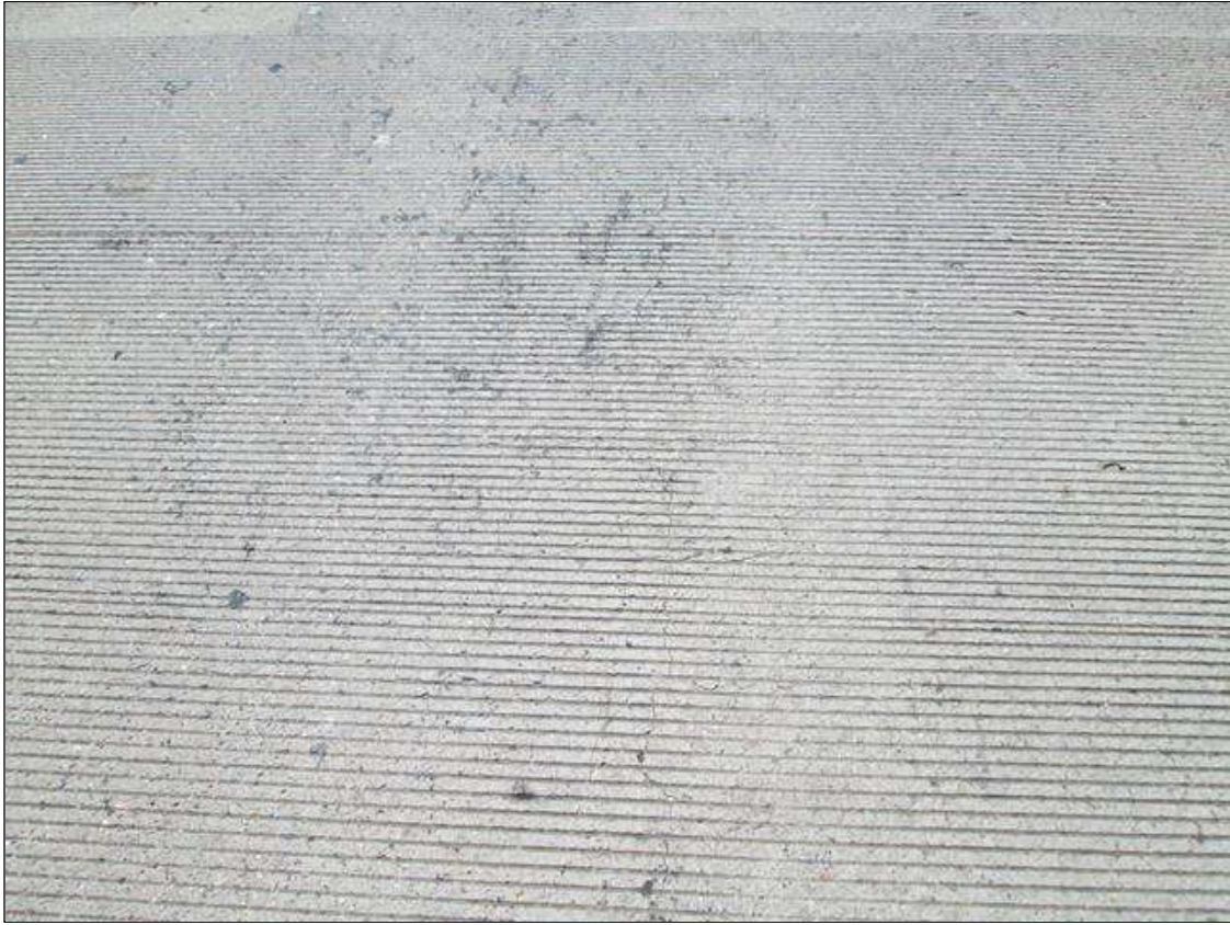
Span 4 Deck: SOME MAP CRACKING AND A FEW TRANSVERSE CRACKS ALSO SOME LONGITUDINAL CRACKS IN EBLs.
