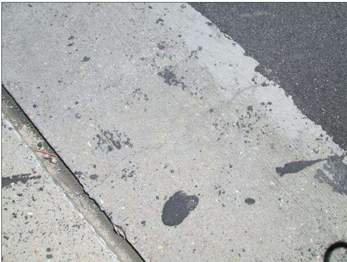
Approach 2: SCATTERED LONGITUDINAL CRACKS ACROSS APPROACH IN EBL AND WBL.
