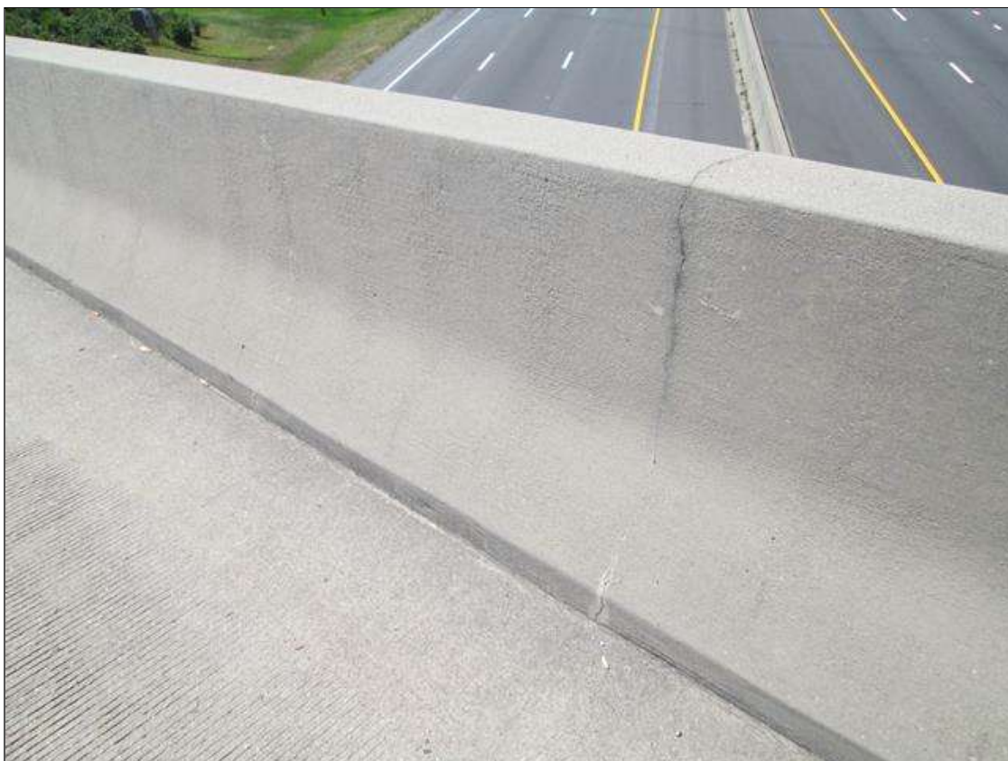
Span 3 Right Bridge Rail: SCATTERED VERTICAL CRACKS WITH EFFLO STAINS
