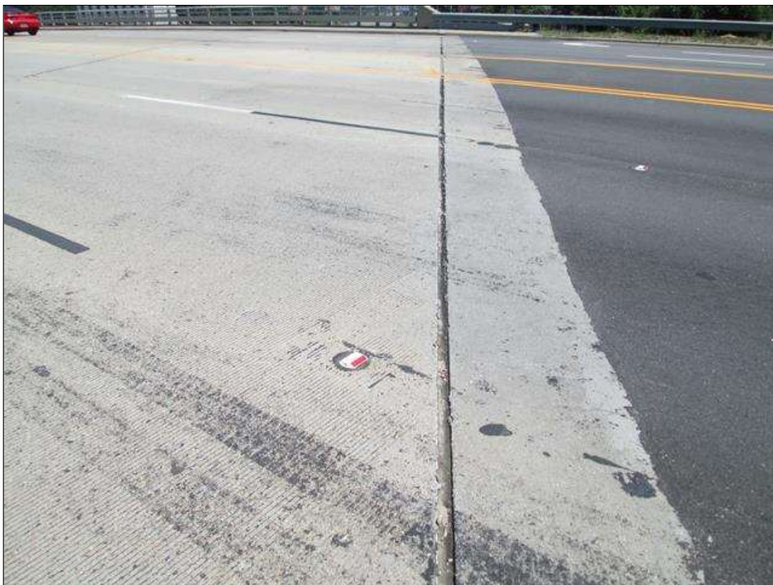
Expansion Joint : DIRT AND SAND AND SMALL GRAVEL INSIDE JOINT OVER END BENT 2.
