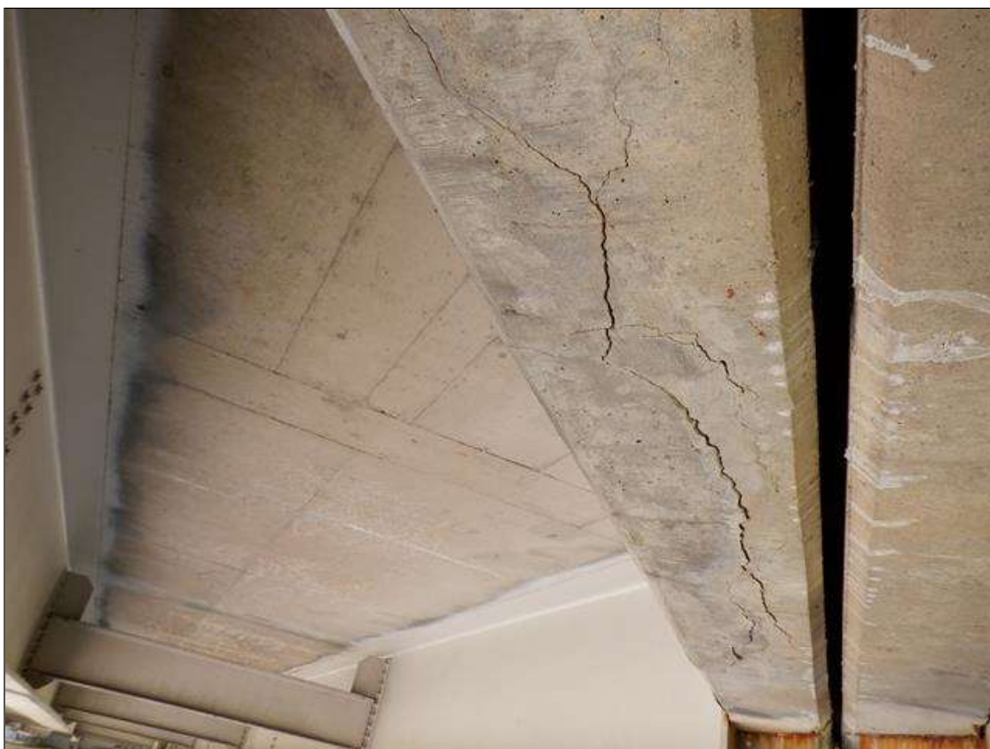
END DIAPHRAGM BAY 2 AT BENT 3: 84" X 10" DELAMINATION
