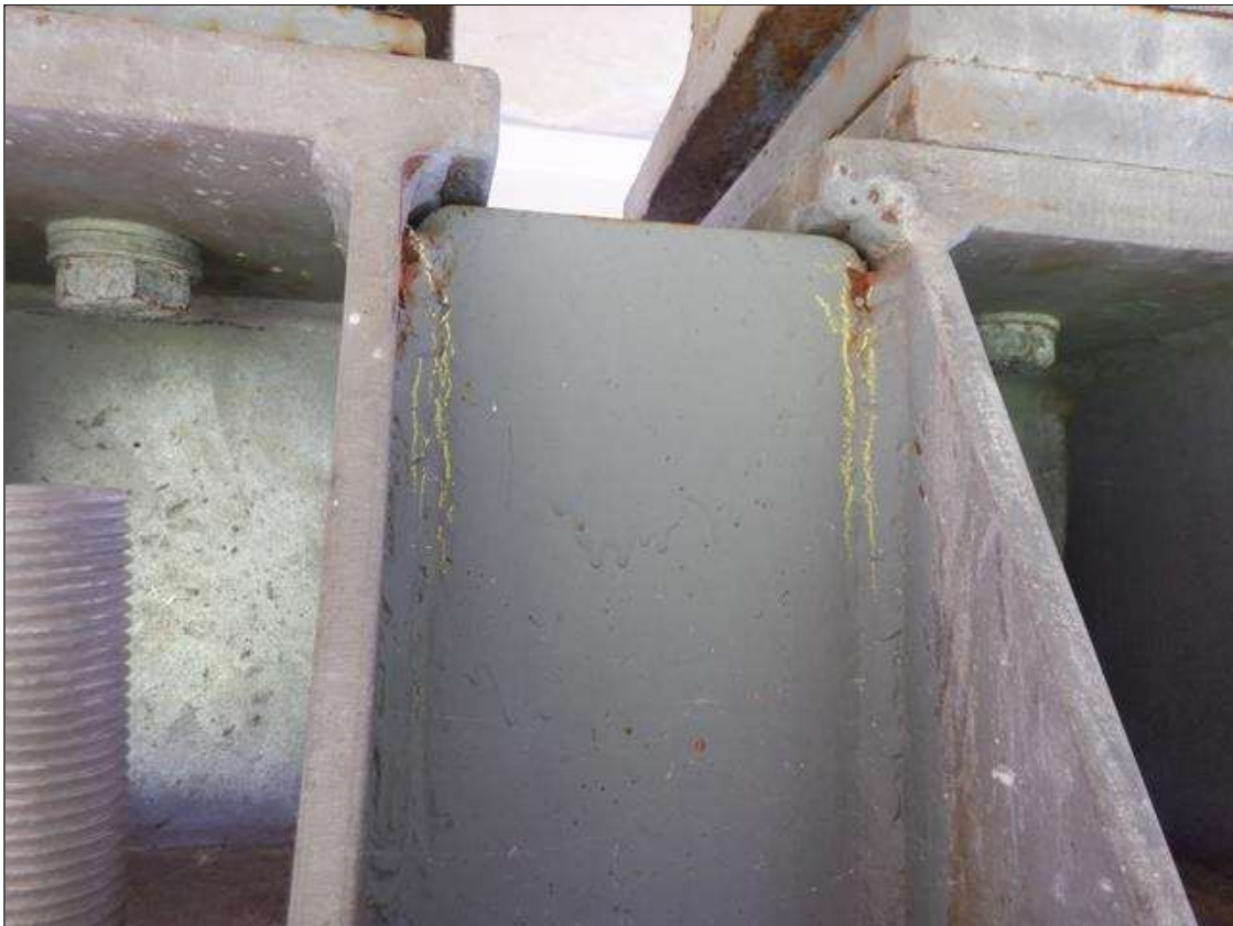
Span 1 Beam 3 Far Bearing: 1" LONG CRACK IN WELD OF WEST STIFFENER TO VERTICAL PLATE (BOTH PLATES) PAR
