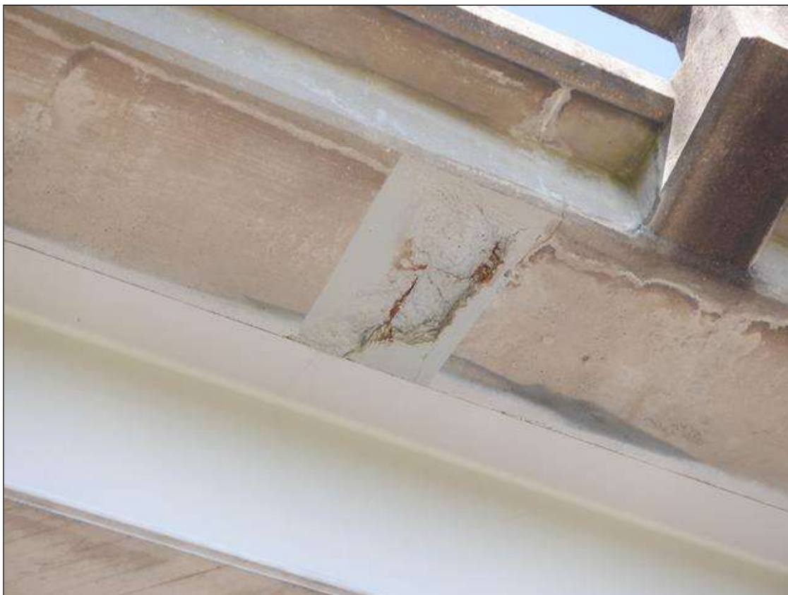
Span 2 Deck: 12" X 6" SPALL IN BOTTOM OF DECK EAST OVERHANG NEAR MIDSPAN OVER TRAFFIC PAR
