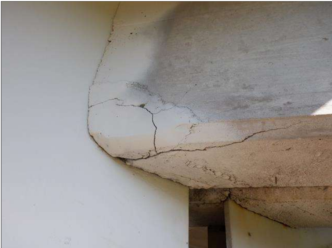
END DIAPHRAGM EAST OVERHANG AT BENT 1: 12" X 4" DELAMINATION
