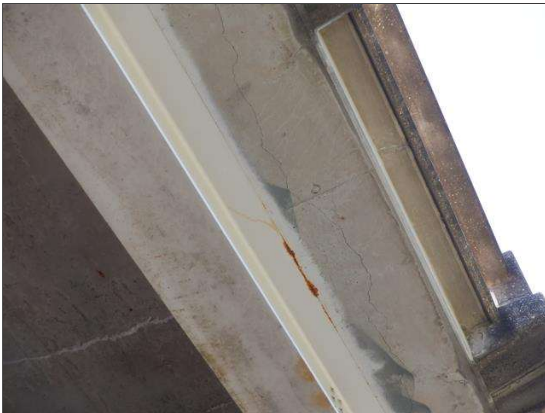
Span 3 Deck: 10 FT OF DELAMINATION IN BOTTOM OF DECK AT WEST OVERHANG NEAR BENT 3
