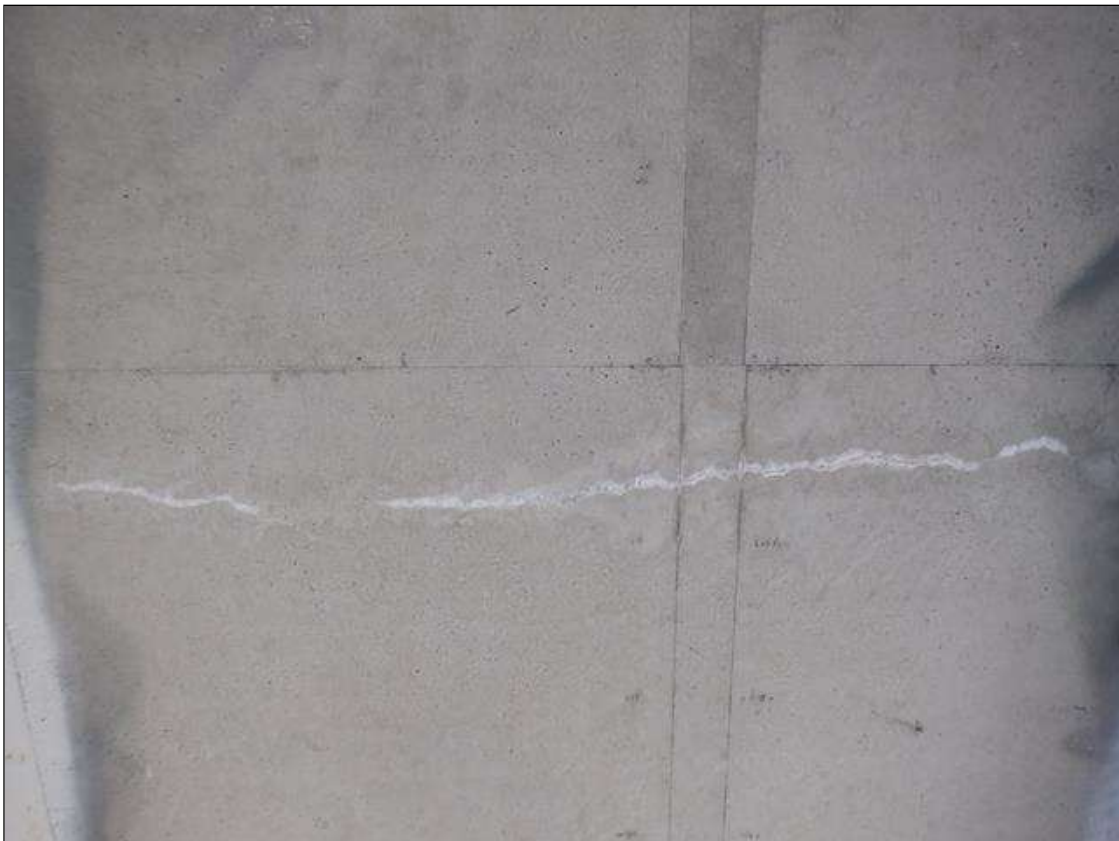
Span 1 Deck: 300 SF. OF TRANSVERSE HAIRLINE CRACKS IN BOTTOM OF DECK
