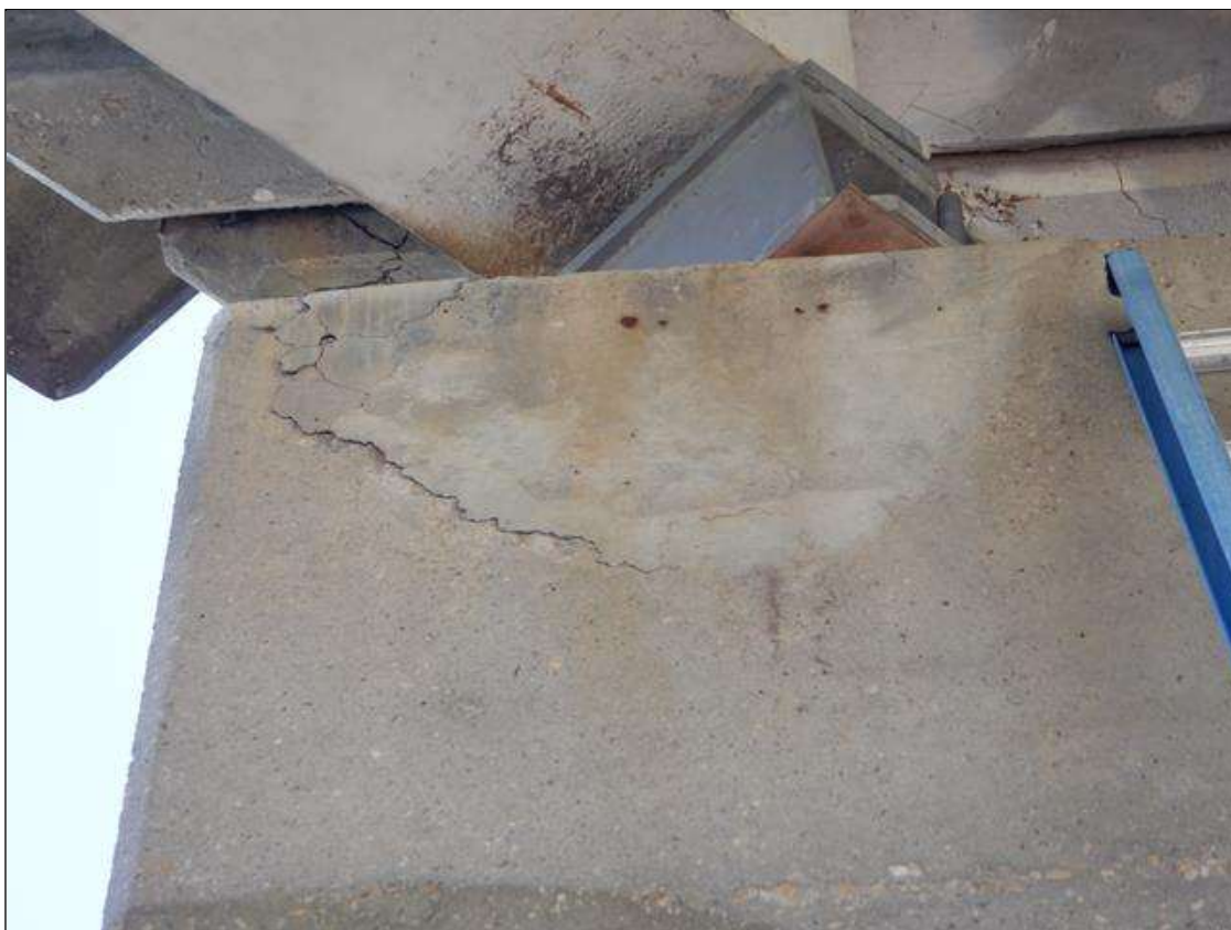
Bent 2 Cap 1: 18" X 6" DELAMINATION IN TOP OF CAP UNDER BEAM 1 SPAN 2 SIDE
