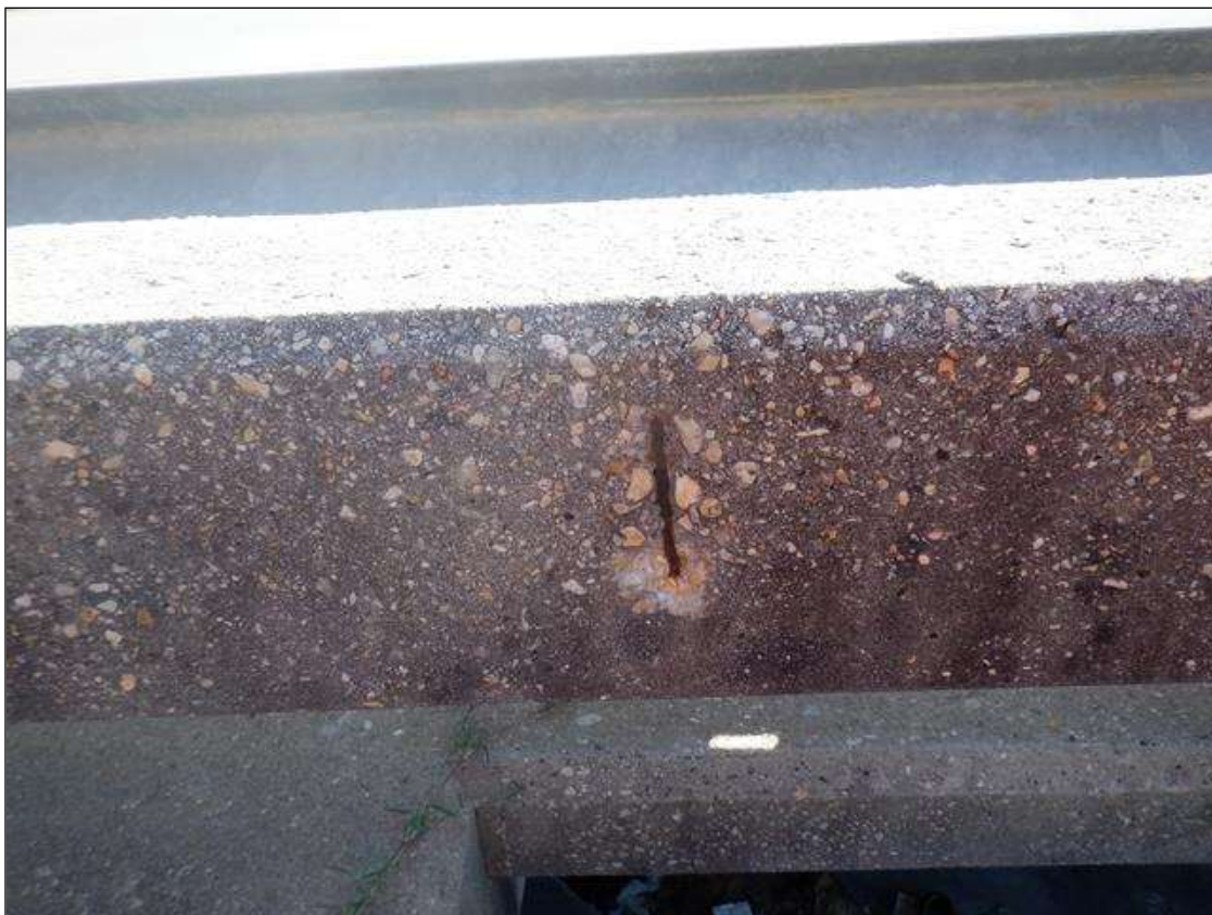
Span 4 Left Bridge Rail: 1 - SPALL WITH EXPOSED REBAR UP TO 6" DIAMETER X 1/2" DEEP IN RAIL
