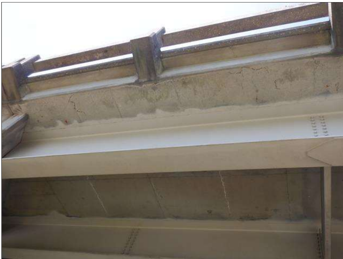
Span 3 Deck: 2-2FTX2FT DELAMINATION IN BOTTOM OF DECK AT EAST OVERHANG NEAR BENT 2 OVER SHOULDER
