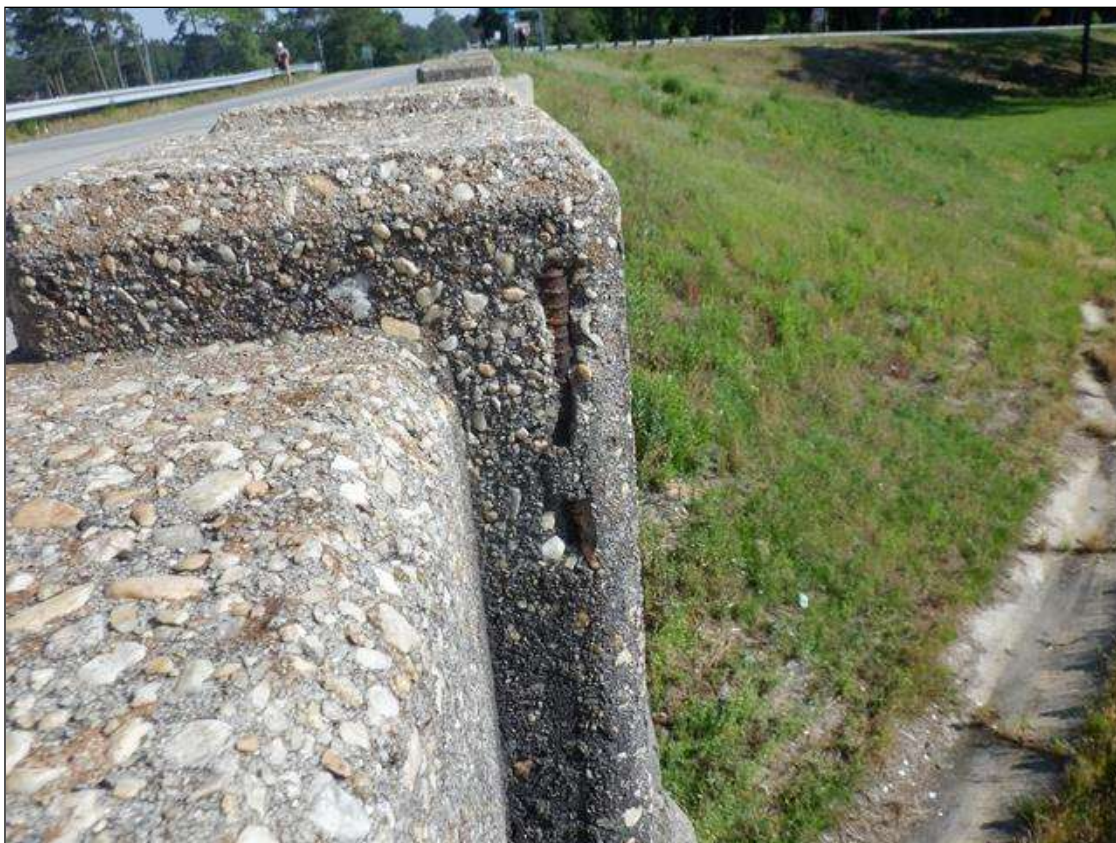
Span 3 Right Bridge Rail: 5 - SPALLS WITH EXPOSED REBAR UP TO 6" DIAMETER X 1/2" DEEP IN RAIL
