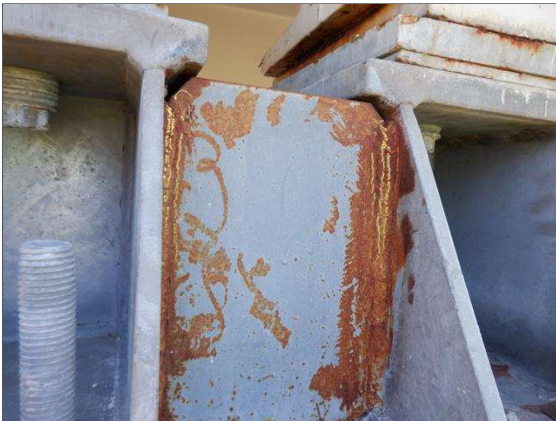
Span 3 Beam 1 Far Bearing: 1" LONG CRACK IN WELD OF EAST STIFFENER TO VERTICAL PLATE (BOTH SIDES) PAR
