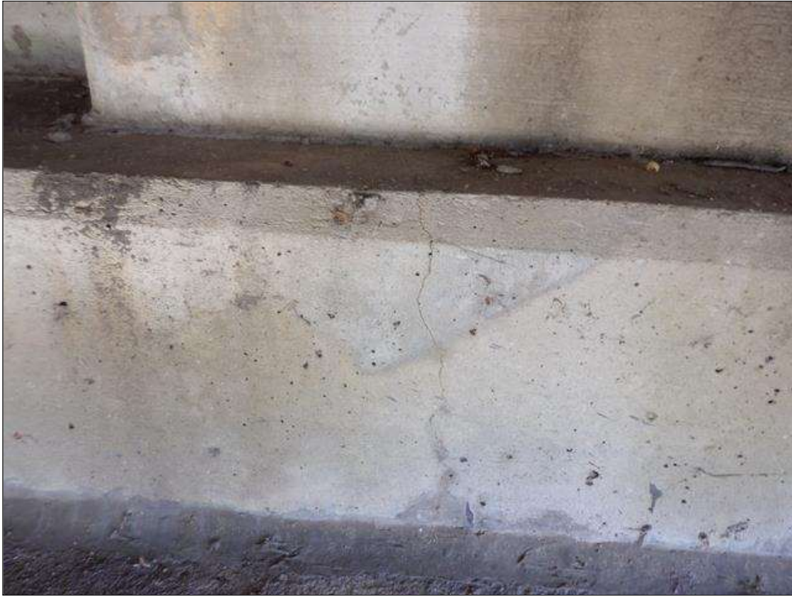
End Bent 1 Cap 1: 3 - 12" VERTICAL CRACKS UP TO 1/16" WIDE UNDER BAY 1
