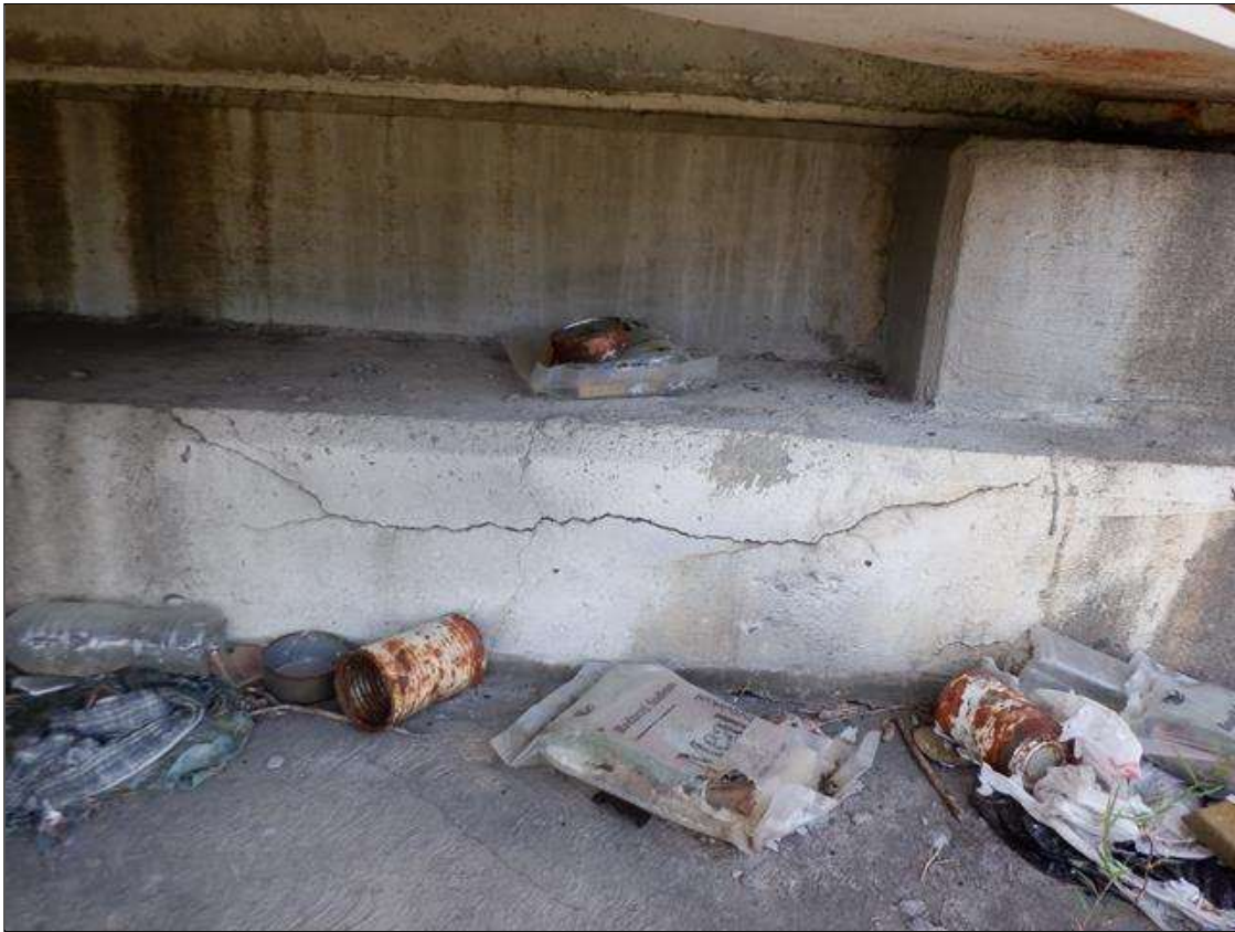
End Bent 2 Cap 1: 36" HORIZONTAL CRACK UP TO 1/8" WIDE UNDER BEAM 4
