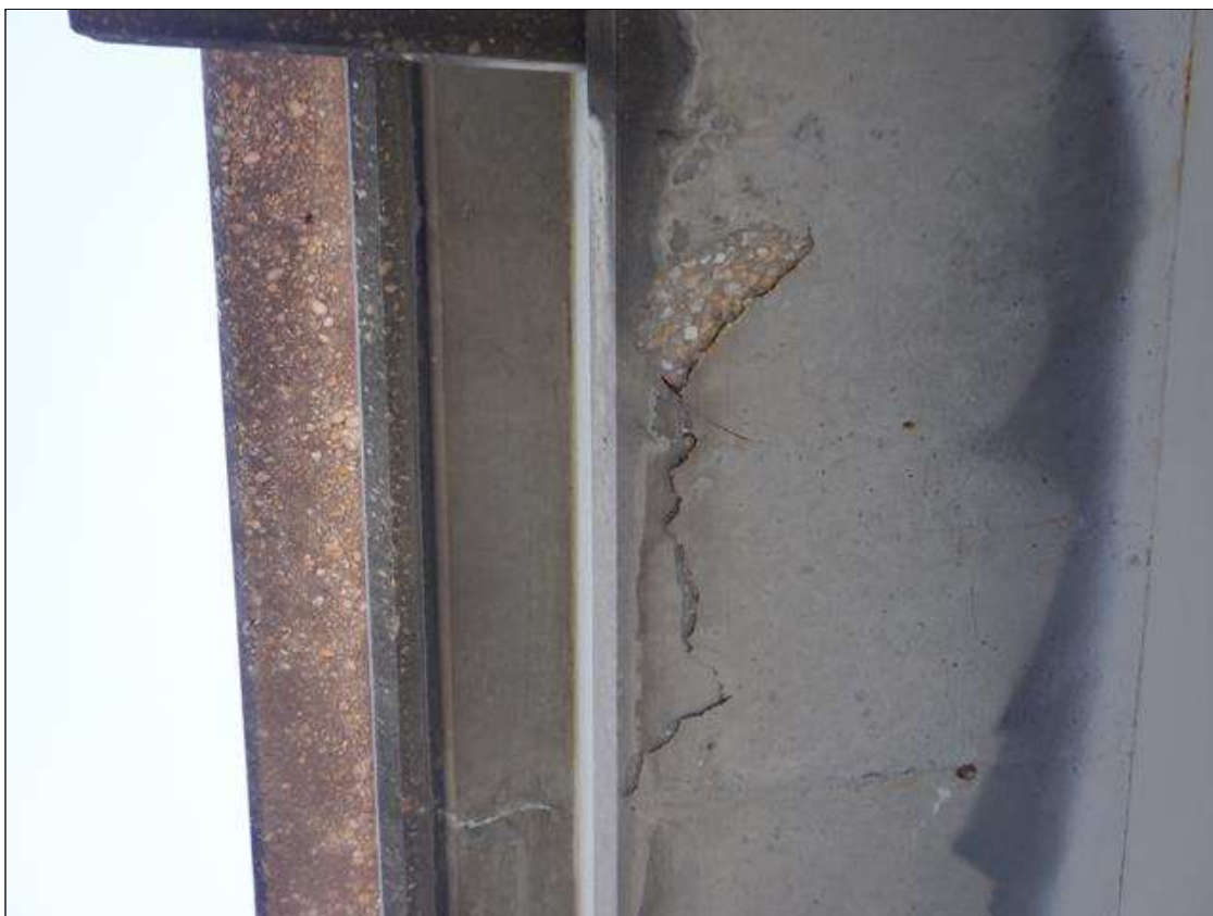
Span 3 Deck: 36" LONG X 12" WIDE DELAMINATION LOCATED UNDER WEST OVERHANG AND OVER THE LEFT SB TRAVEL LANE
