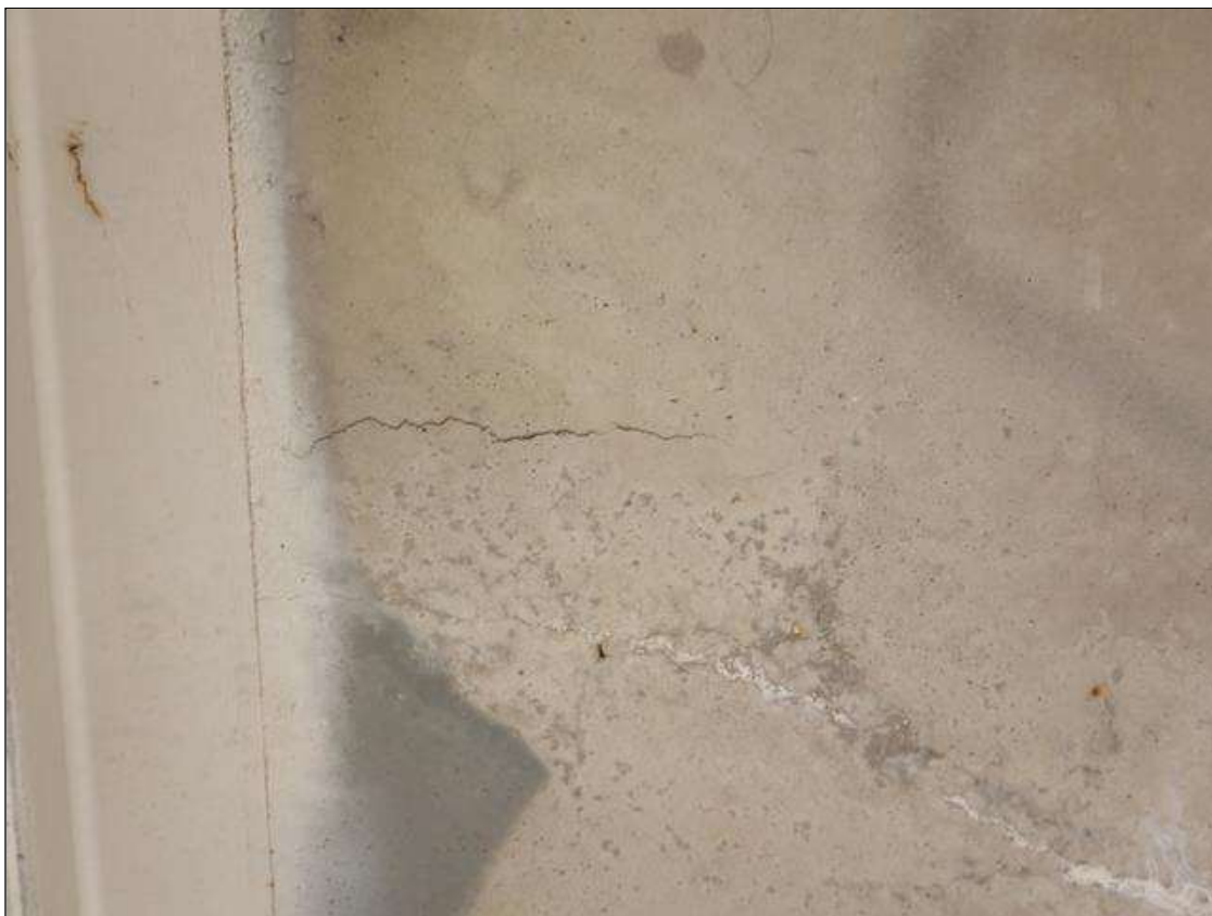
Span 3 Deck: 2 SF DELAMINATION LOCATED IN BOTTOM OF DECK BAY 1 OVER CENTERLINE OF SB TRAVEL LANES
