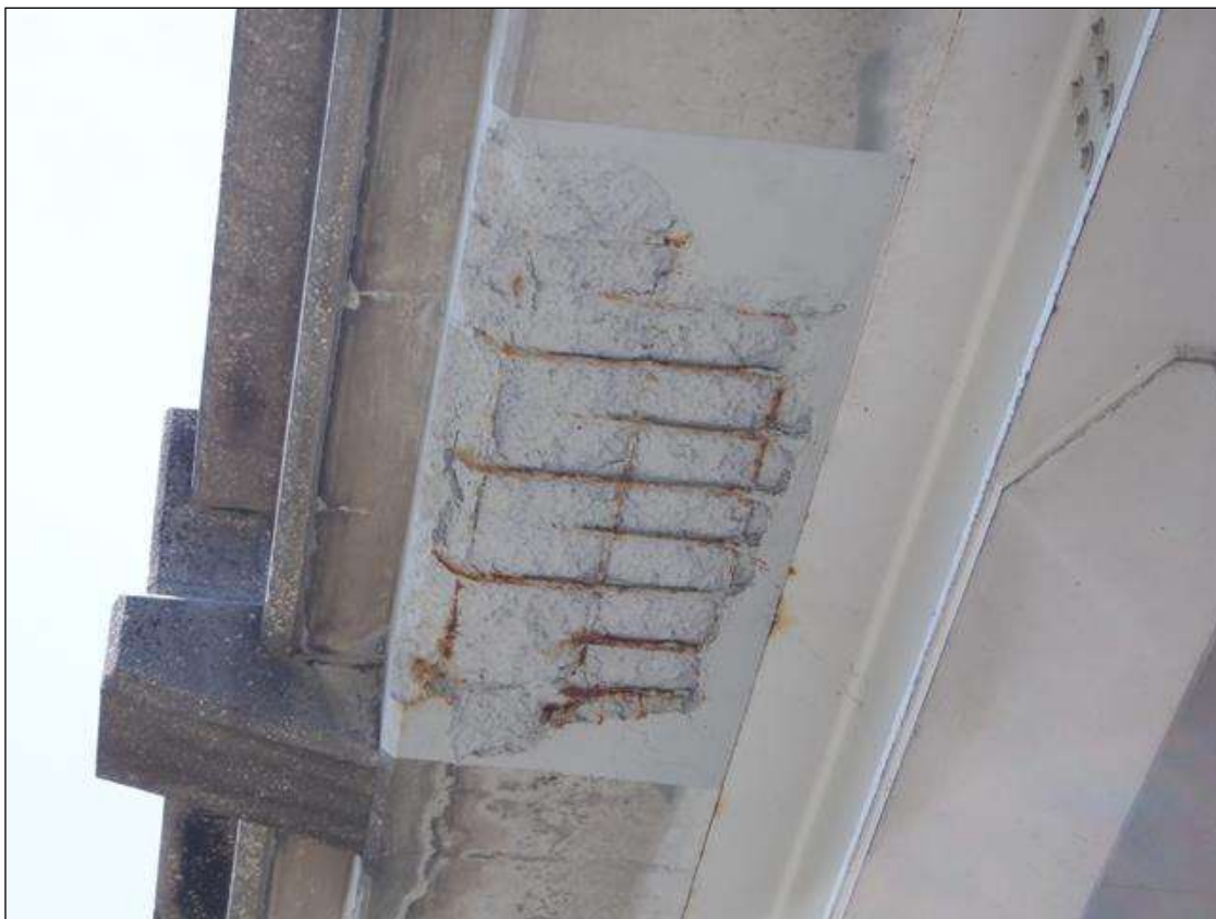
Span 3 Deck: 48" X 24" X 2" SPALL WITH EXPOSED REBAR IN BOTTOM OF DECK EAST OVERHANG OVER TRAFFIC PAR
