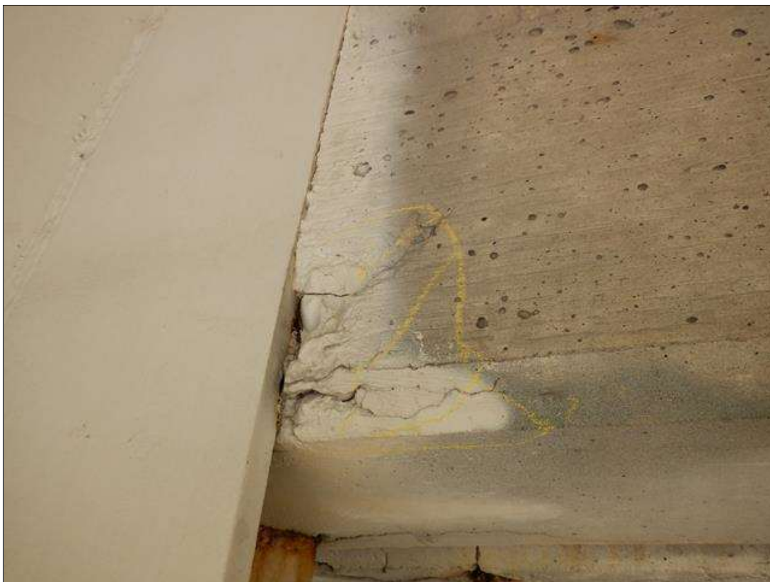
END DIAPHRAGM BAY 2 AT BENT 2: 2 - 6" DIAMETER DELAMINATIONS
