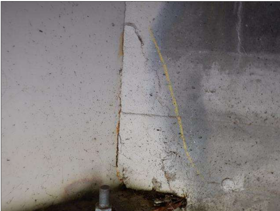
End Bent 1 Abutment/Backwall : 12" X 6" DELAMINATION IN BAY 1
