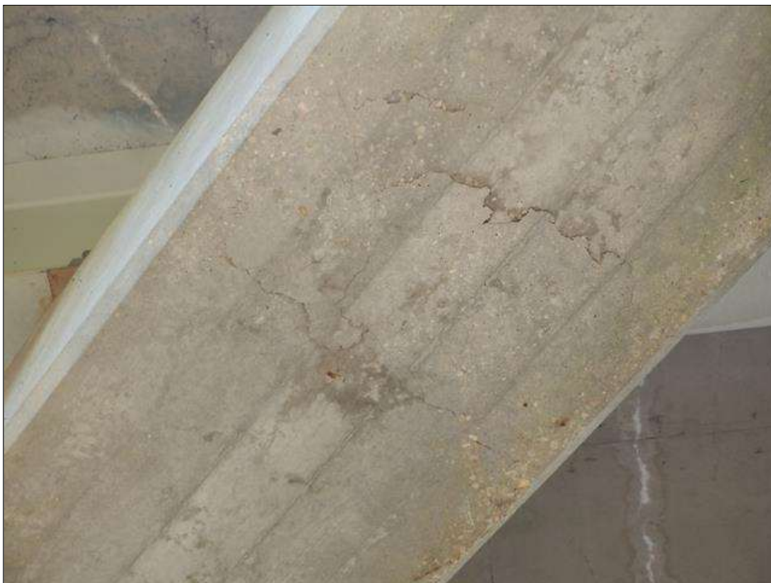
Bent 1 Cap 1: 24" DIAMETER DELAMINATION IN BOTTOM OF CAP BETWEEN COLUMNS 2 AND 3
