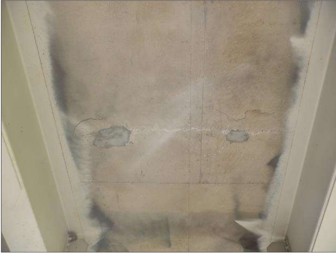
Span 1 Deck: 2 - 12" DIAMETER DELAMINATIONS IN BOTTOM OF DECK 20 FT. FROM BENT 1 BAY 3
