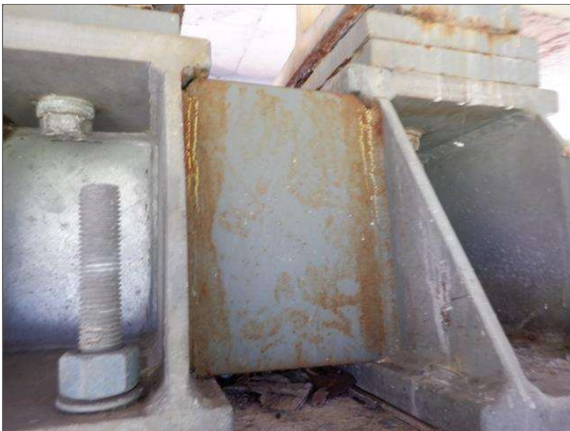
Span 4 Beam 2 Near Bearing: 2" LONG CRACK IN WELD OF EAST STIFFENER TO VERTICAL PLATE PAR
