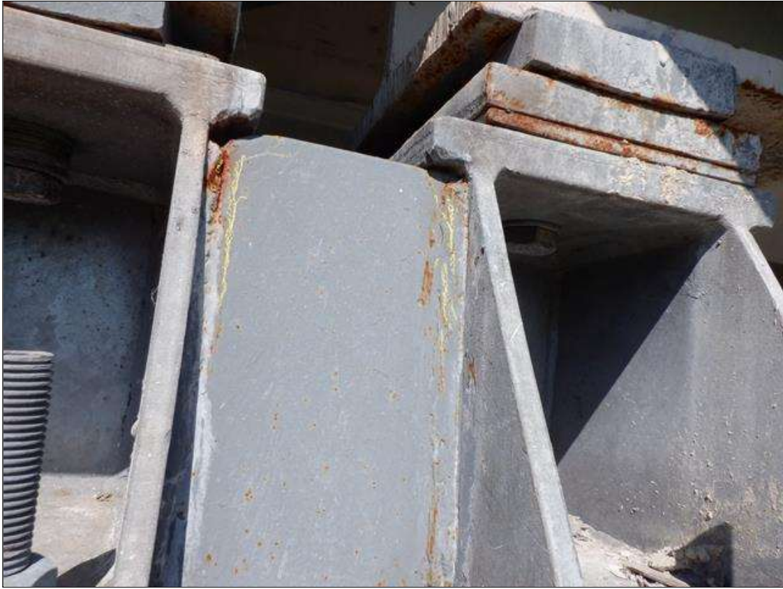
Span 1 Beam 4 Far Bearing: 1" LONG CRACK IN WELD OF EAST STIFFENER TO VERTICAL PLATE (BOTH PLATES) PAR
