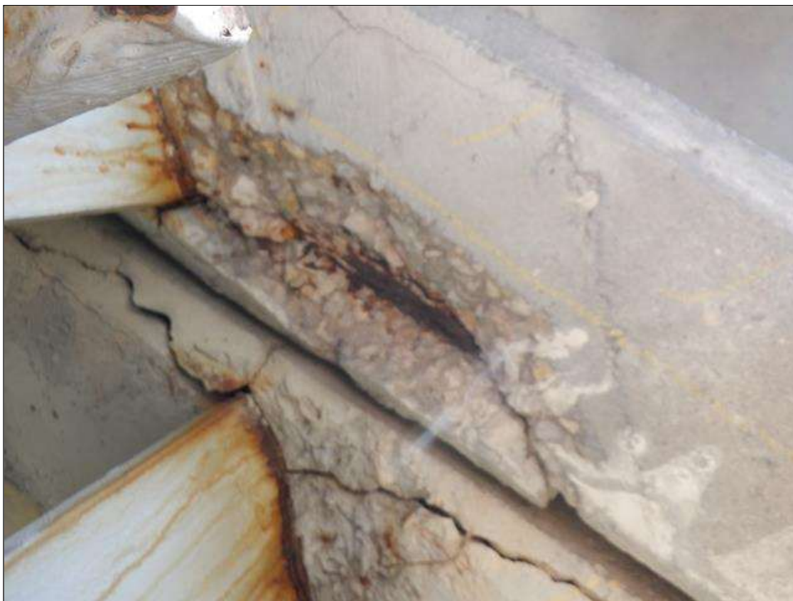
END DIAPHRAGM EAST OVERHANG AT BENT 2: 14" X 3" X 2" DEEP SPALL WITH EXPOSED REBAR
