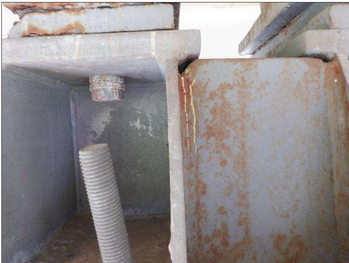
Span 2 Beam 3 Far Bearing: 1" LONG CRACK IN WELD OF WEST STIFFENER TO VERTICAL PLATE (BOTH SIDES) PAR
