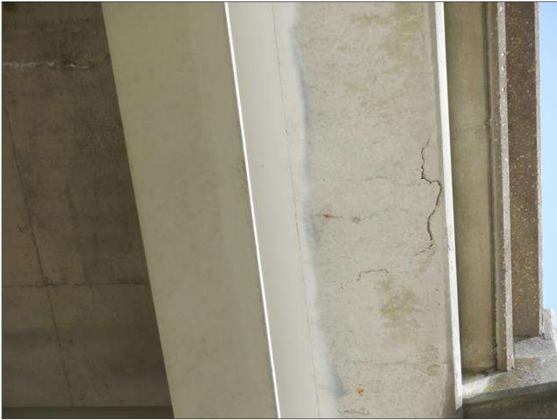
Span 3 Deck: 2 SF DELAMINATION LOCATED 12 FT FROM BENT 2 UNDER EAST OVERHANG OVER LEFT SHOULDER OF SB TRAVEL LANE
