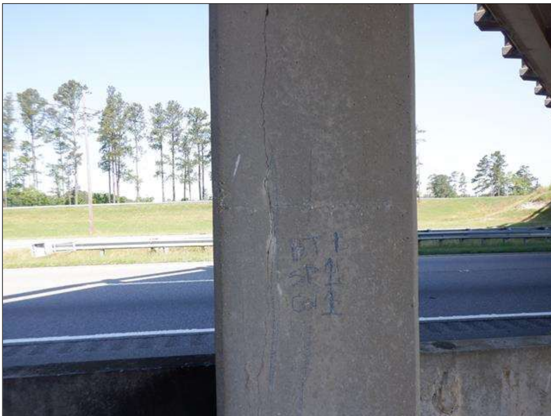
Bent 1 Pile 1: 96" X 6" DELAMINATION IN SOUTH FACE
