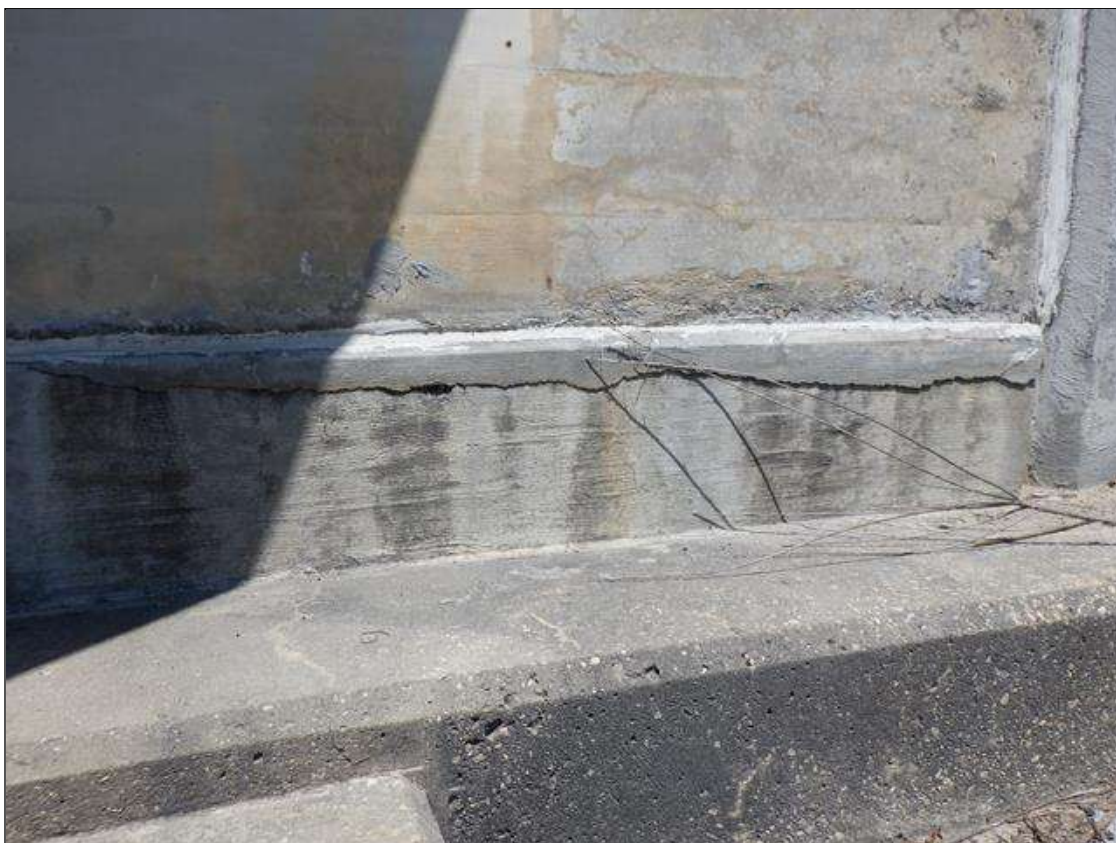
End Bent 2 Abutment/Backwall : 3 SF. OF HAIRLINE MAP CRACKING UNDER EAST OVERHANG WITH 4FT X 1/16" HORIZONTAL CRACK
