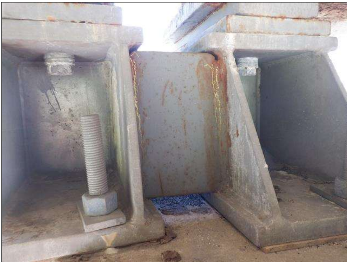
Span 2 Beam 1 Far Bearing: 1" LONG CRACK IN WELD OF EAST STIFFENER TO VERTICAL PLATE (BOTH PLATES) PAR
