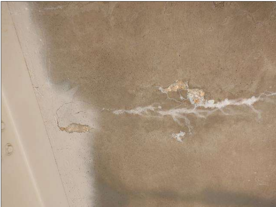
Span 4 Deck: 2FT LONG X 8' WIDE X 1/2" DEEP SPALL LOCATED IN BAY 3 BOTTOM OF DECK
