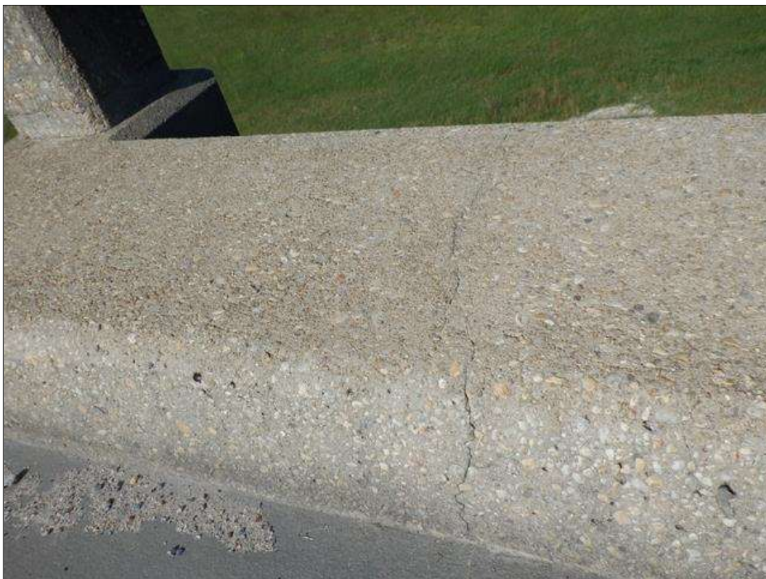
Span 4 Left Bridge Rail: 8 - 18" TRANSVERSE CRACKS UP TO 1/16" WIDE IN CURB
