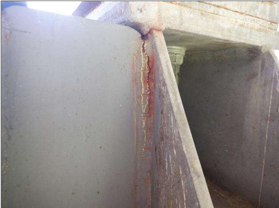
Span 1 Beam 1 Far Bearing: 2" LONG CRACK IN WELD OF EAST STIFFENER TO VERTICAL PLATE PAR
