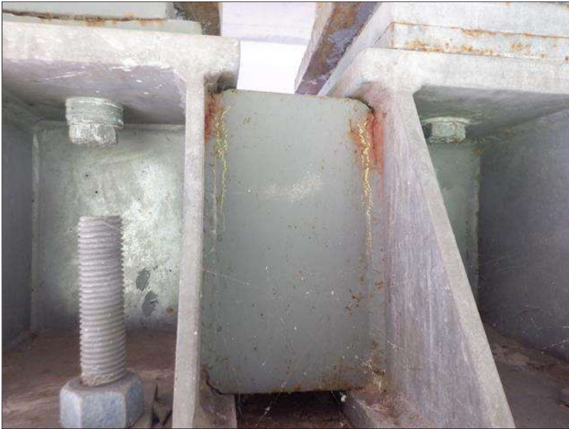
Span 1 Beam 2 Far Bearing: 2" LONG CRACK IN WELD OF EAST STIFFENER TO VERTICAL PLATE (BOTH PLATES) PAR
