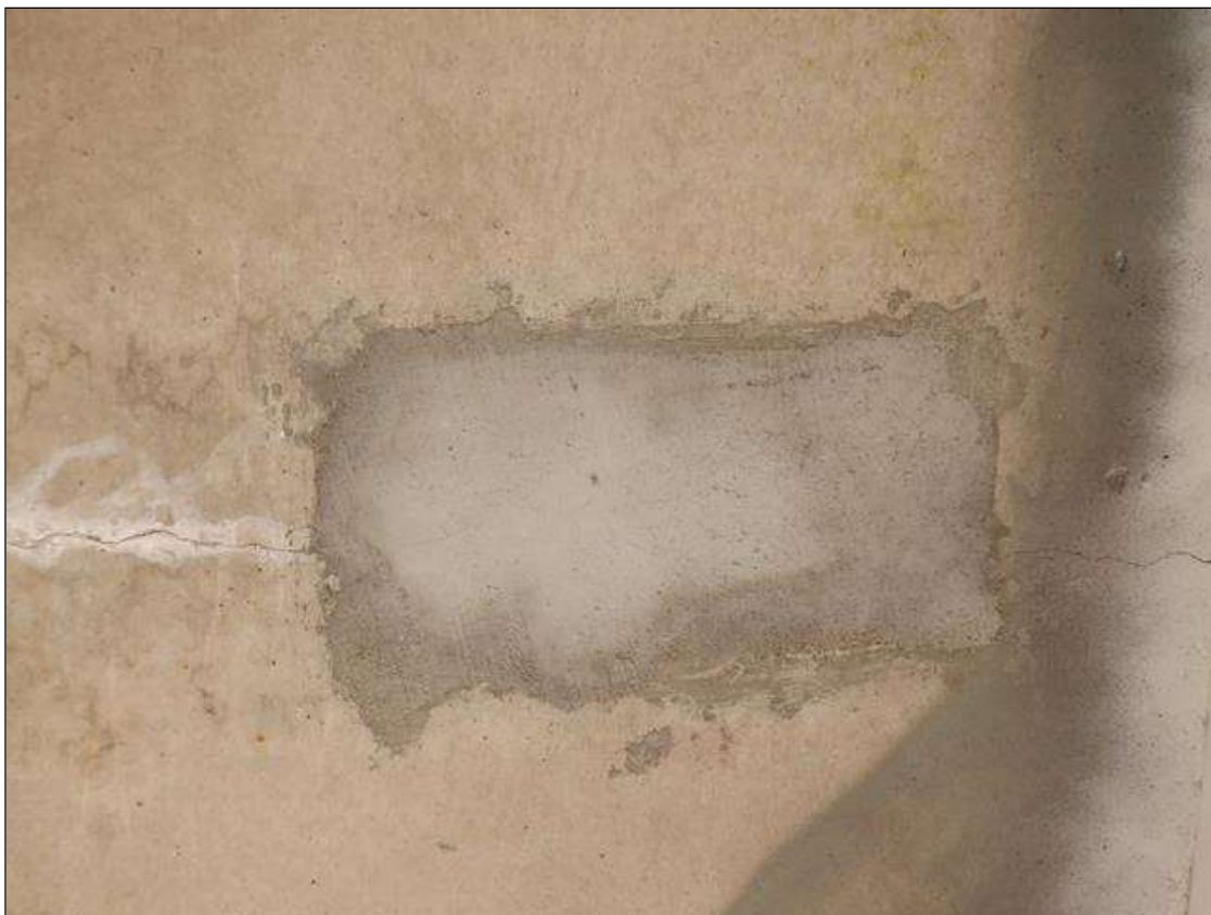
Span 1 Deck: 25 SF. OF PATCHED AREAS IN BOTTOM OF DECK
