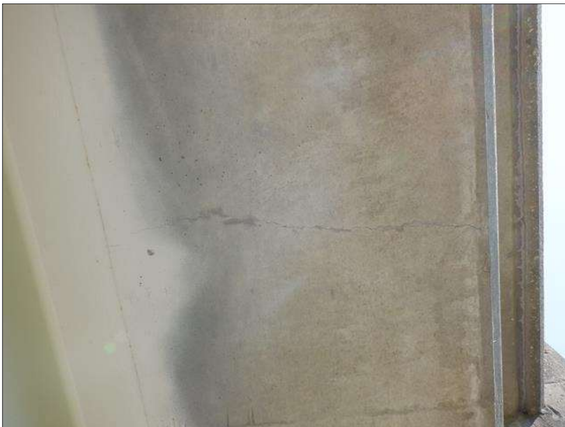
Span 1 Deck: 14 - 24" TRANSVERSE HAIRLINE CRACKS IN BOTTOM OF DECK EAST OVERHANG
