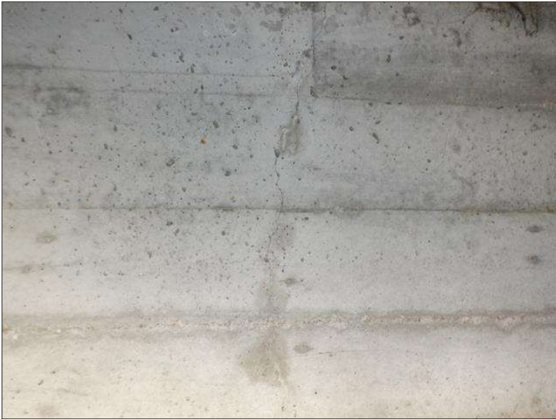
End Bent 1 Abutment/Backwall : 3 - 24" VERTICAL HAIRLINE CRACKS IN BAY 1
