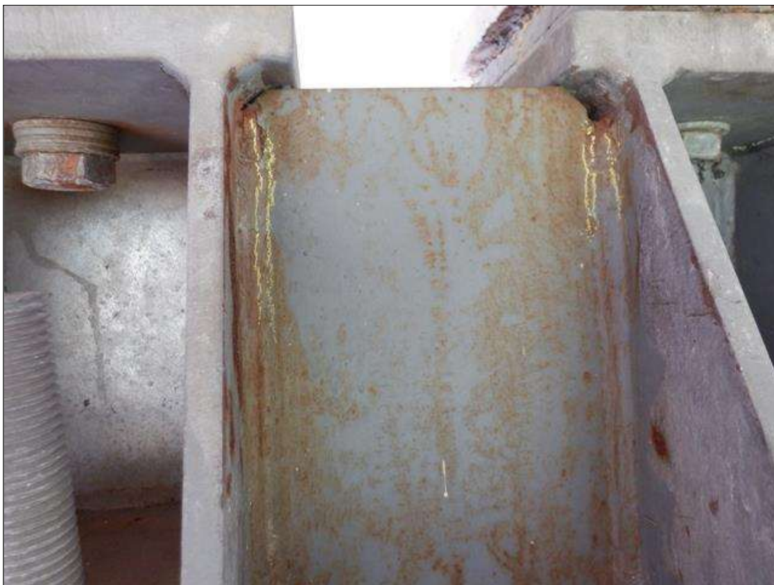
Span 4 Beam 3 Near Bearing: 1" LONG CRACK IN WELD OF WEST STIFFENER TO VERTICAL PLATE PAR
