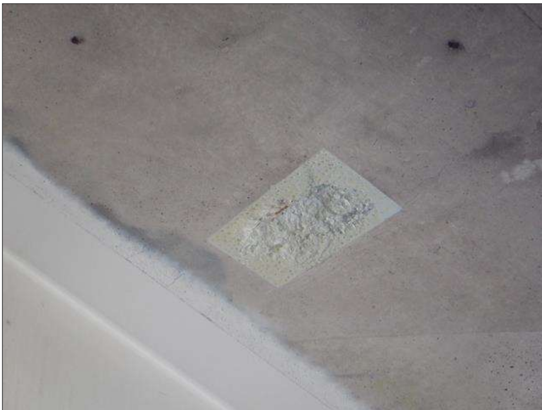
Span 2 Deck: 12" DIAMETER SPALL IN BOTTOM OF DECK BAY 1 OVER TRAFFIC PAR
