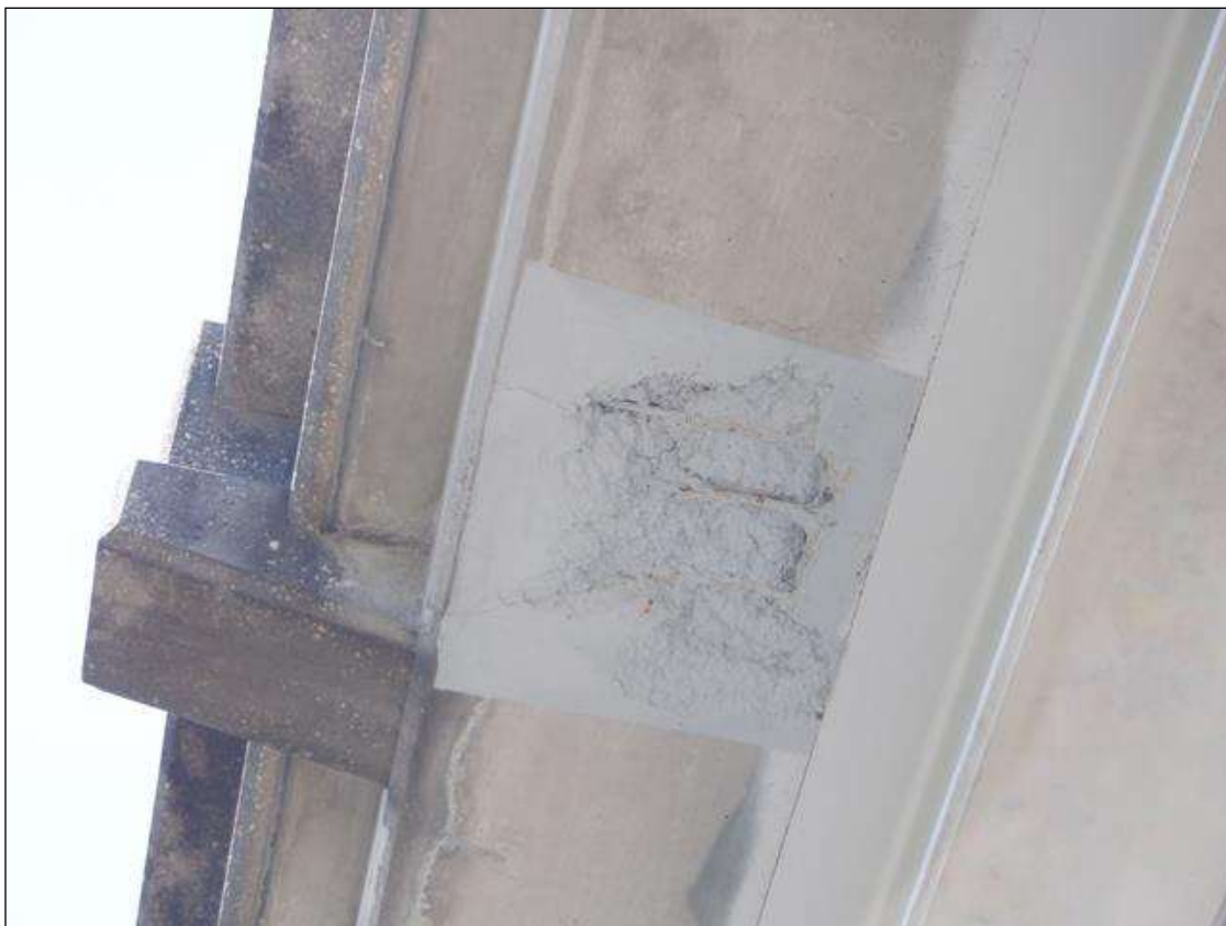
Span 2 Deck: 12" DIAMETER SPALL IN BOTTOM OF DECK EAST OVERHANG OVER TRAFFIC PAR
