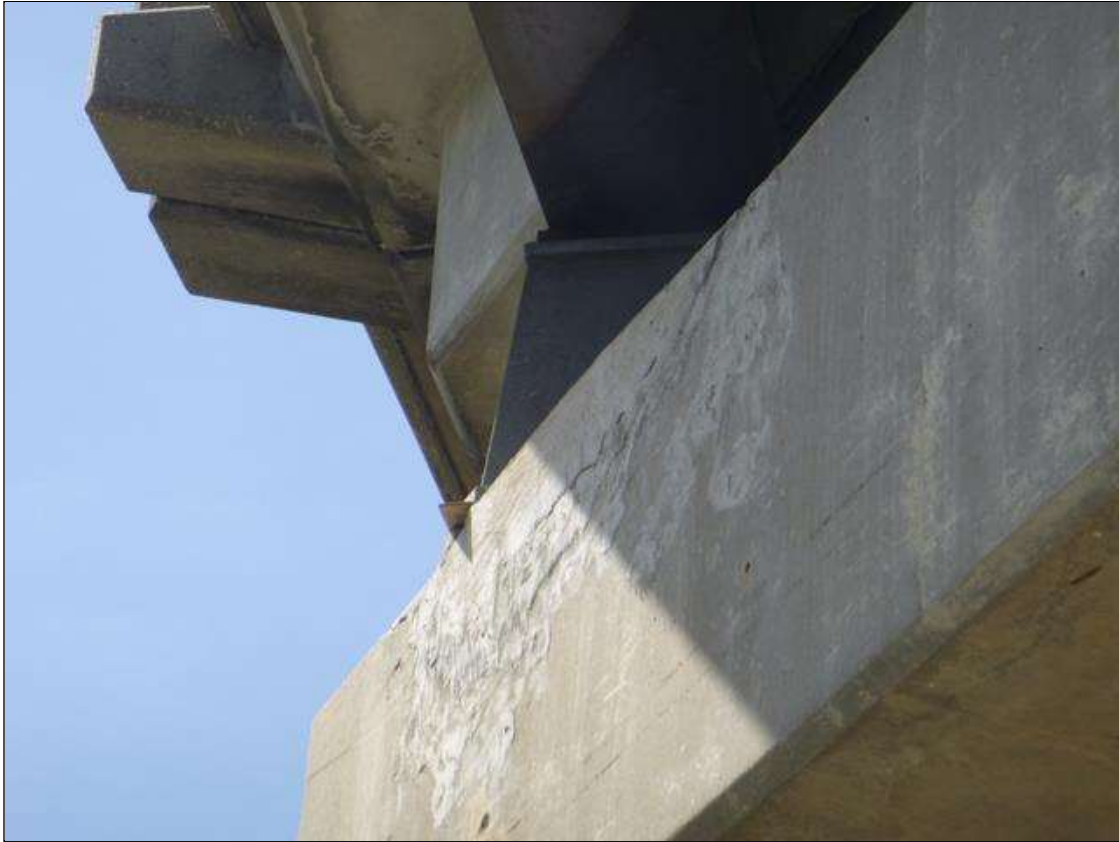
Bent 1 Cap 1: 3' X 8" PATCHED AREA, TOP OF EAST FACE BELOW BEAM 4.
