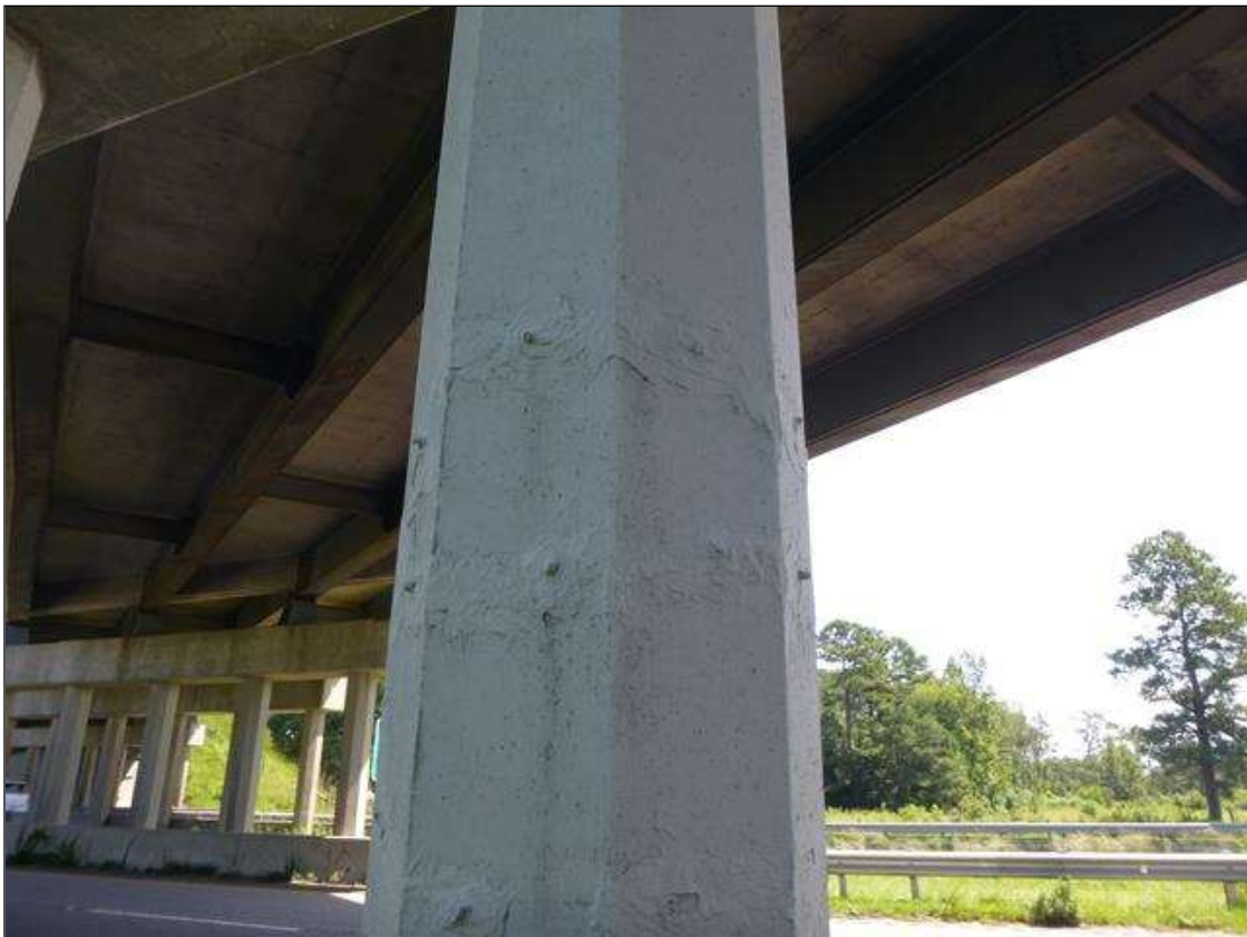
Bent 1 Pile 2: EPOXY SEALED CRACKS THROUGHOUT AT MID HEIGHT.
