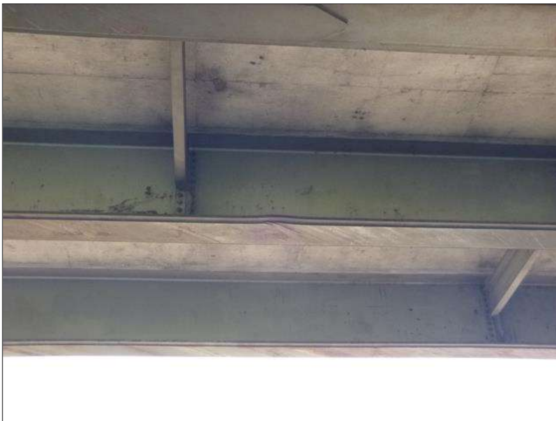
Span 2 Beam 3: (2) 2" GOUGES UP TO 1/2" DEEP, BOTTOM OF COVER PLATE, CAUSING UPWARD DEFLECTION OF BOTTOM FLANGE UP TO 1", 2' WEST OF FIRST INTERMEDIATE DIAPHRAGM.
