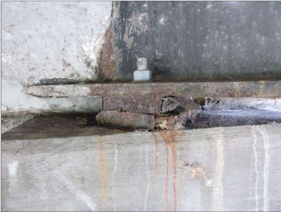
Span 1 Beam 1 Near Bearing: BEARING ASSEMBLY HAS RUST SCALE, BEAM 1.
