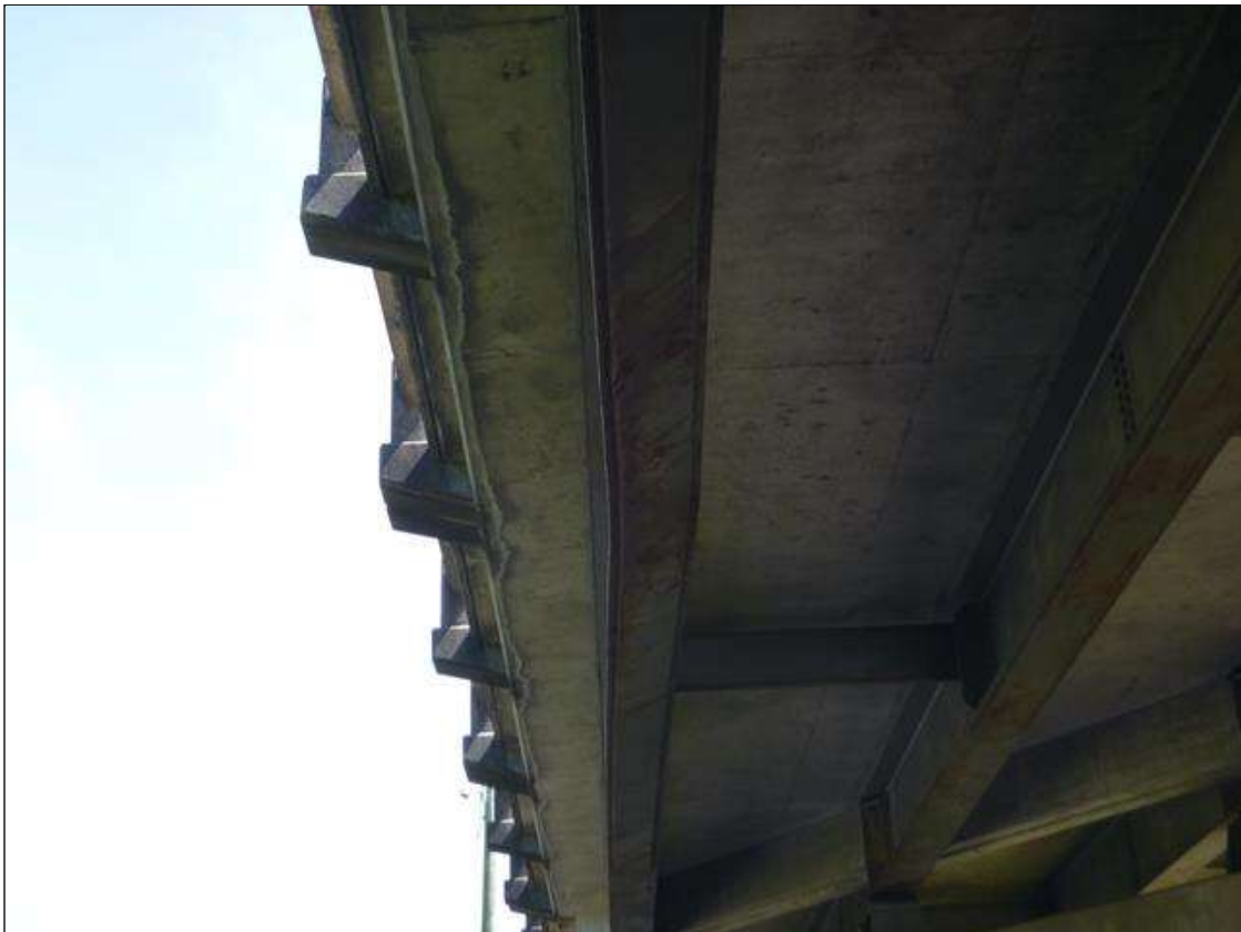
Span 2 Beam 1: 15 Feet of Damage: Bottom flange is bent 2" south over I-95 southbound lane.
