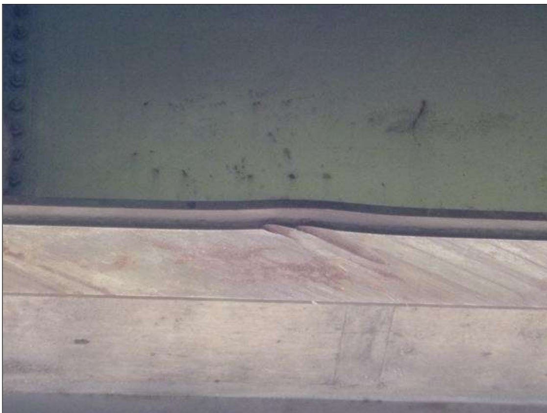
Span 2 Beam 3: (2) 2" GOUGES UP TO 1/2" DEEP, BOTTOM OF COVER PLATE, CAUSING UPWARD DEFLECTION OF BOTTOM FLANGE UP TO 1", 2' WEST OF FIRST INTERMEDIATE DIAPHRAGM.
