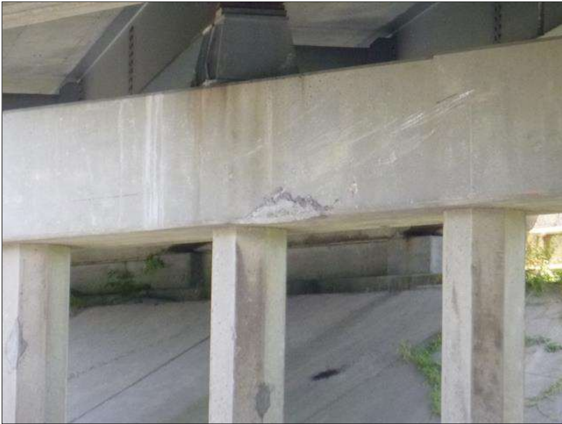
Bent 4 Cap 1: LOWER SIDE OF THE CAP BETWEEN PILES 3-4, WEST FACE, LOWER CORNER, APPROX 3SQFT UNSOUND PATCHING (HAIRLINE MAP CRACKED)
