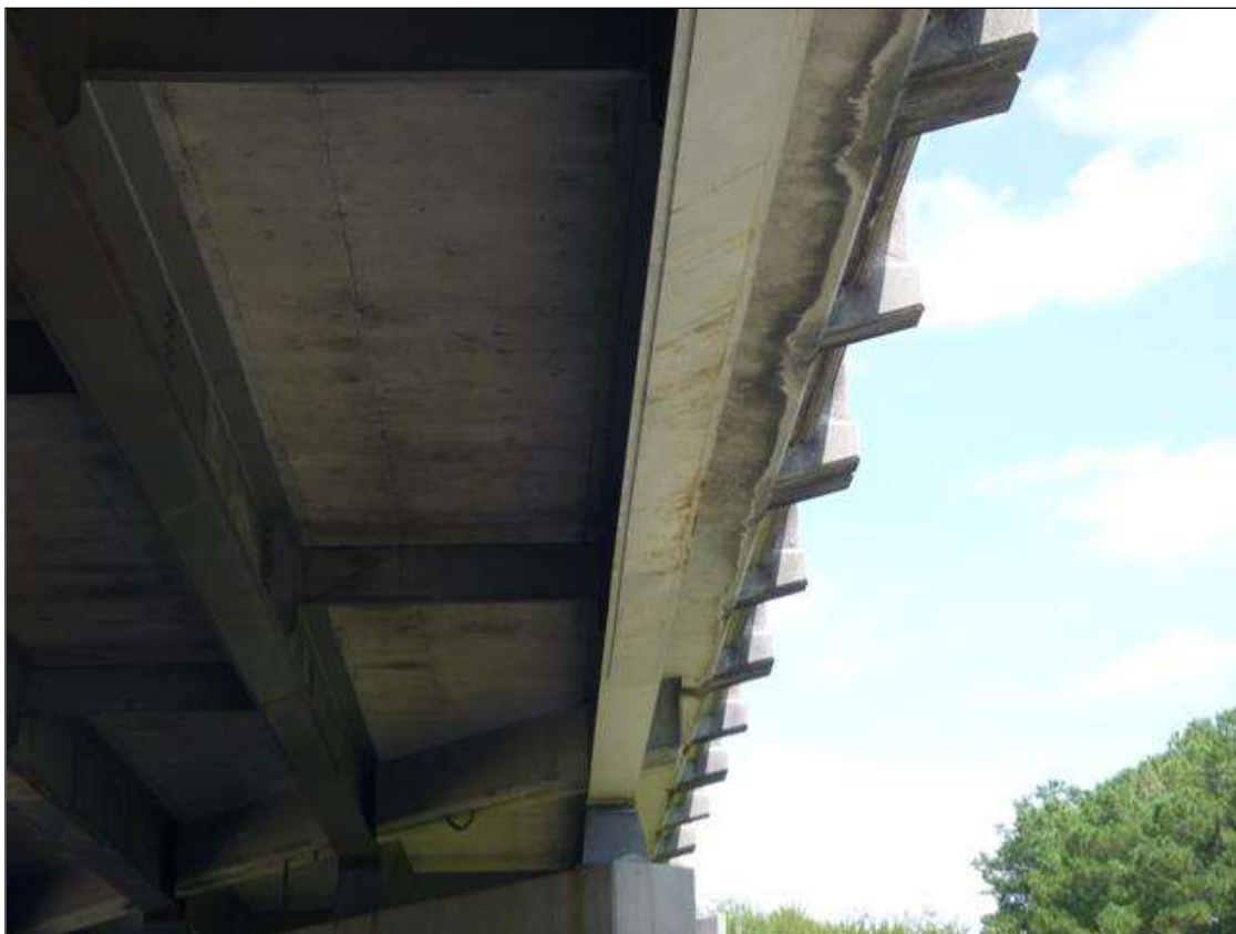
Span 4 Beam 4: 6' OF SCRAPES AND SHALLOW GOUGES ALONG UNDERSIDE OF BOTTOM FLANGE, NEAR MIDSPAN.
