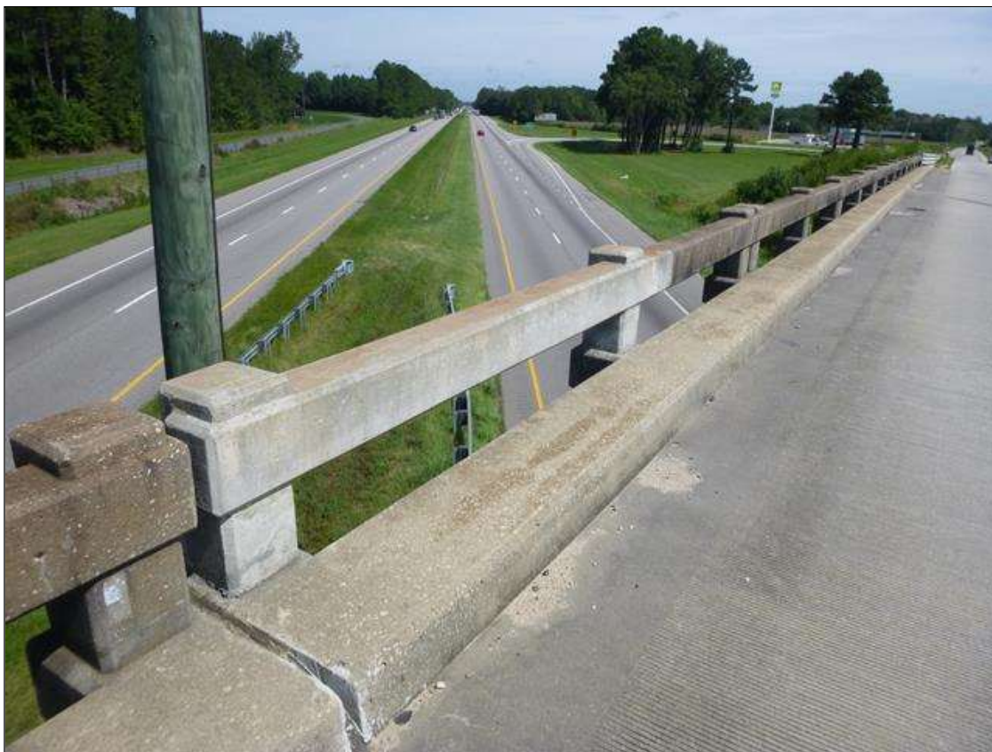
Span 4 Left Bridge Rail: 11' REPAIR TO RAIL BEGINNING AT BENT 3.
