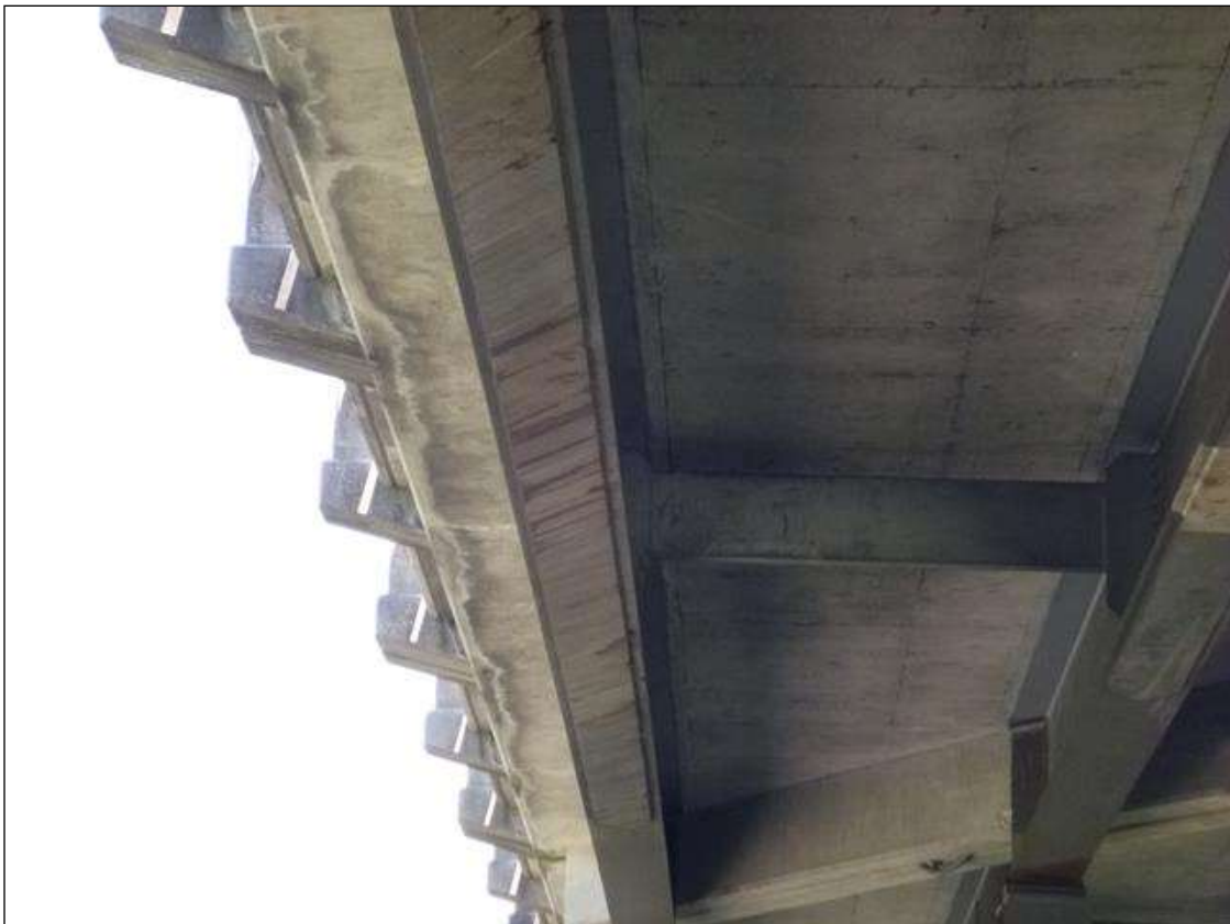
Span 4 Beam 1: 20' OF SCRAPES ALONG UNDERSIDE OF BOTTOM FLANGE, AT MIDSPAN.
