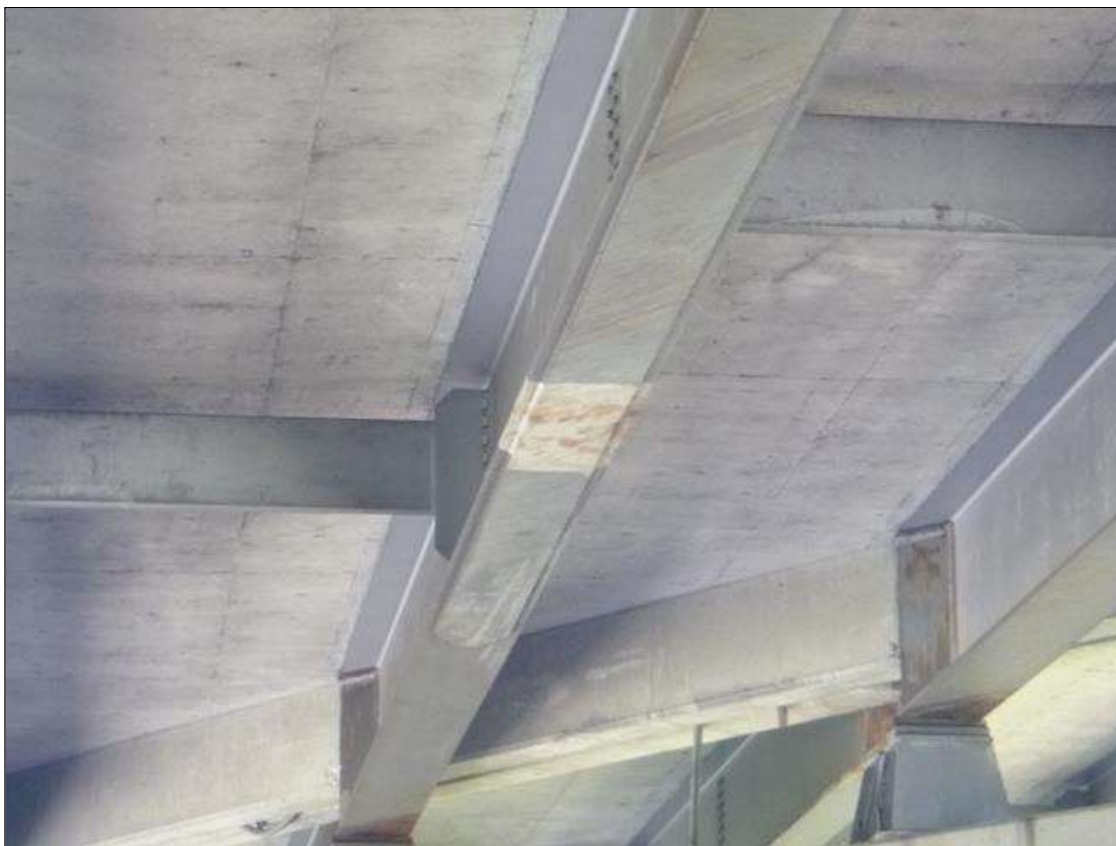
Span 4 Beam 2: NEAR MID SPAN, PAST IMPACT DAMAGE REPAIR
