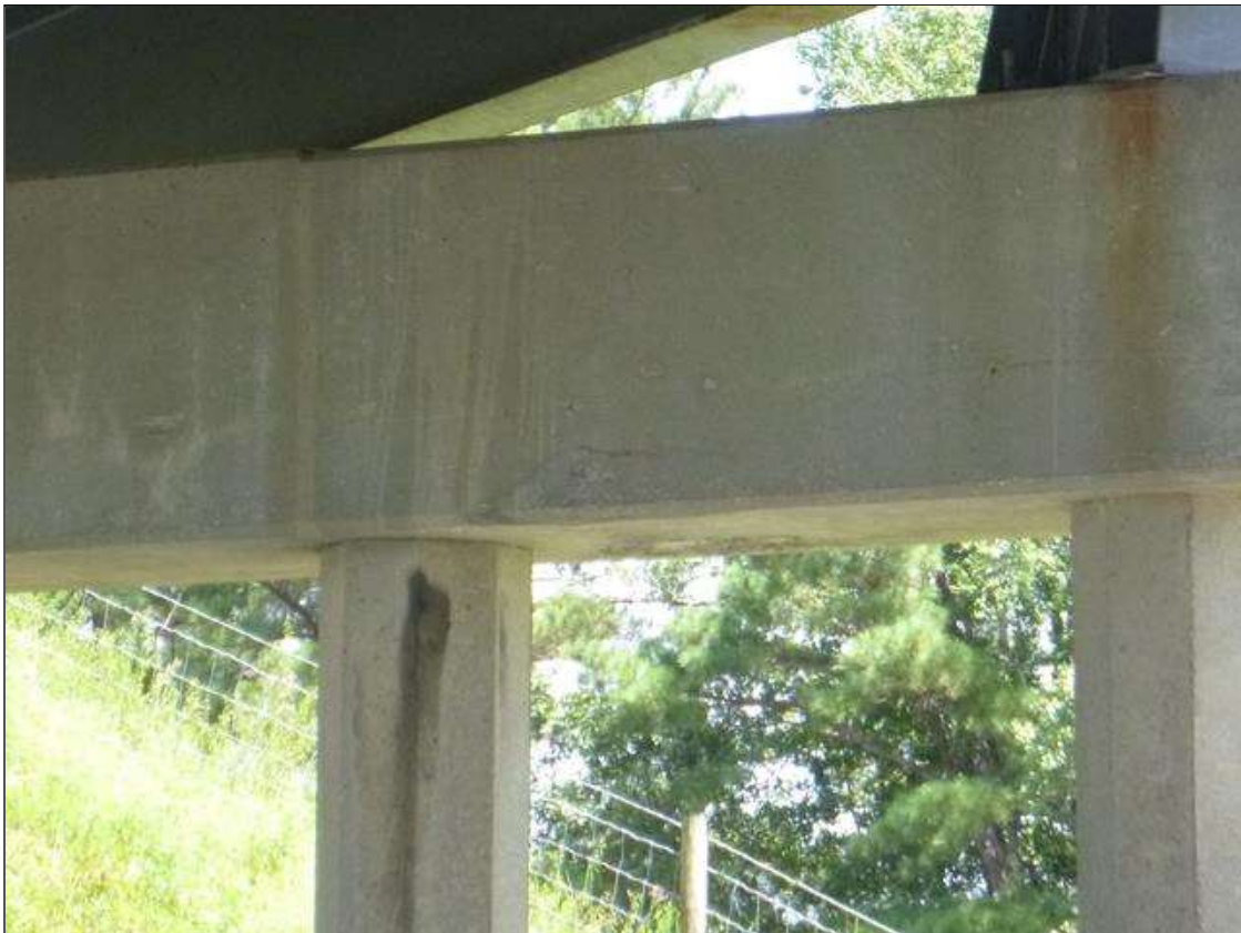
Bent 4 Cap 1: LOWER SIDE OF THE CAP BETWEEN PILES 3-4, EAST FACE, LOWER CORNER, LONGITUDINAL CRACKING UP TO 1/8"
