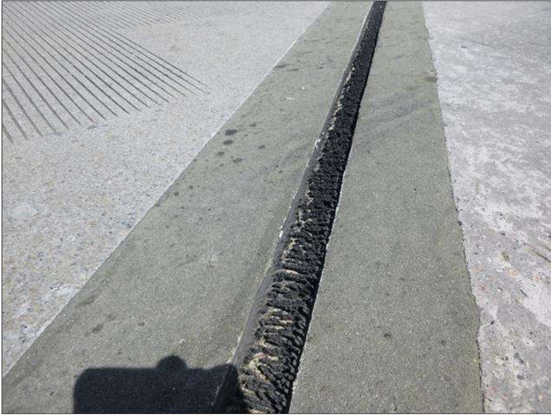
Expansion Joint, End Bent 2 : TOP OF THE SEAL, DEGRADATION AND SURFACE CRACKING ALONG THE LENGTH
