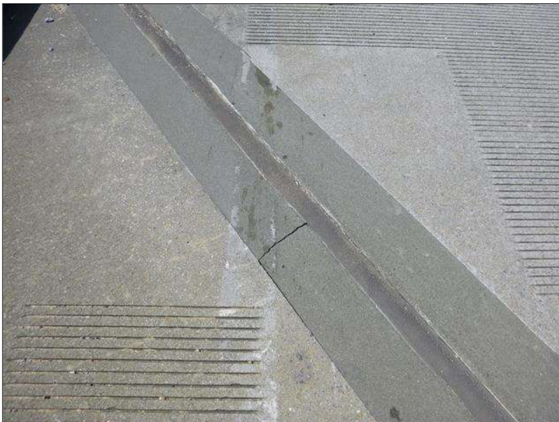
Expansion Joint, Bent 4 : EASTBOUND LANE, TRANSVERSE CRACKING IN THE ADJACENT DECK HEADER UP TO 1/32".
