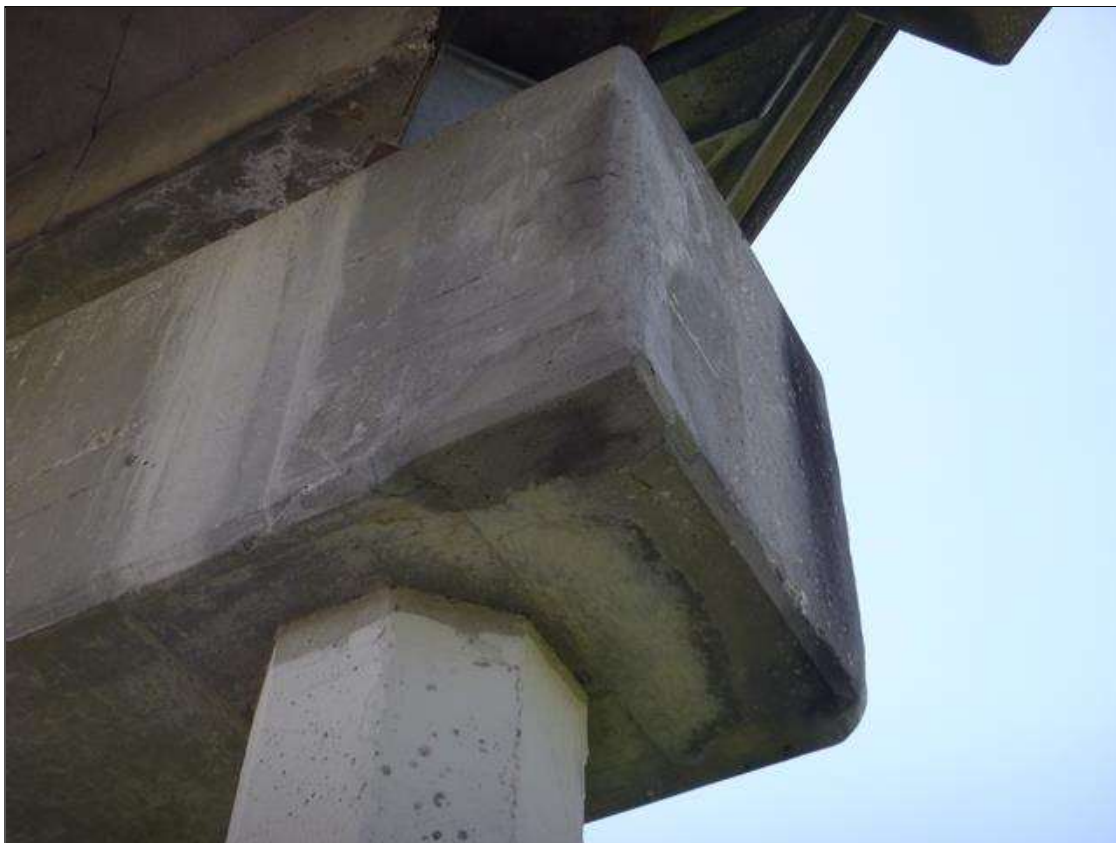
Bent 1 Cap 1: 14" X 6" X 6" PATCHED AREA, BOTTOM CORNER OF EAST FACE AT NORTH END.
