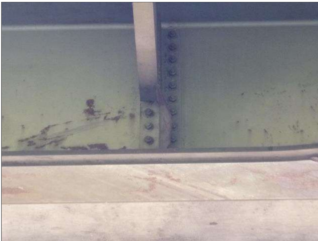
Span 2 Beam 3: Intermediate Diaphragm: BOTTOM HALF OF GUSSET PLATE IS BENT AND DISTORTED ON NORTH SIDE OF BEAM.
