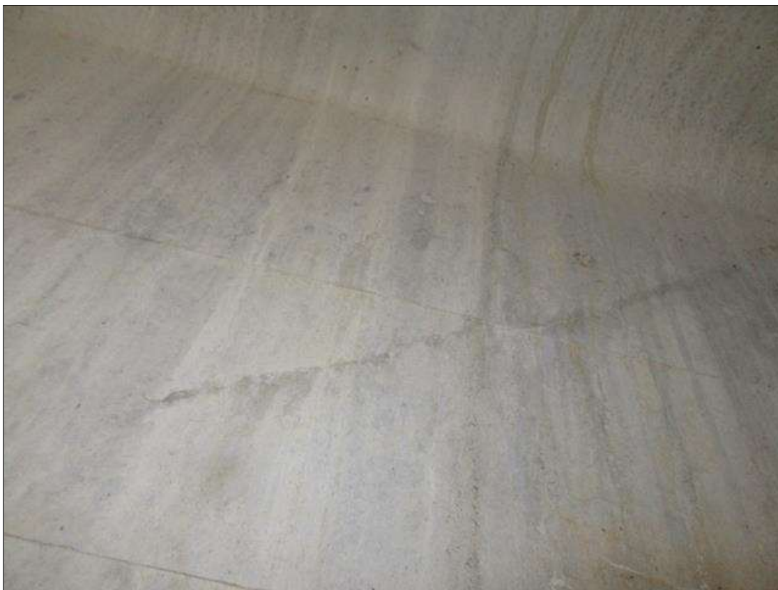
Span 2 Beam 1: 1- 2 ' LONG X HAIRLINE DIAGONAL SHEER CRACKING IN WEB BAY 1 SIDE AT FAR END
