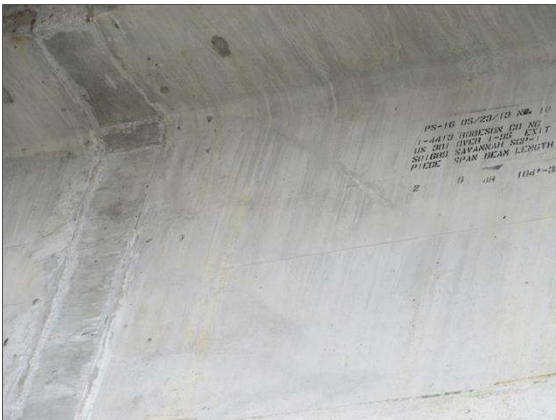
Span 2 Beam 4: 1- 2' LONG X HAIRLINE DIAGONAL SHEER CRACKING IN WEB AT RIGHT SIDE AT NEAR END.
