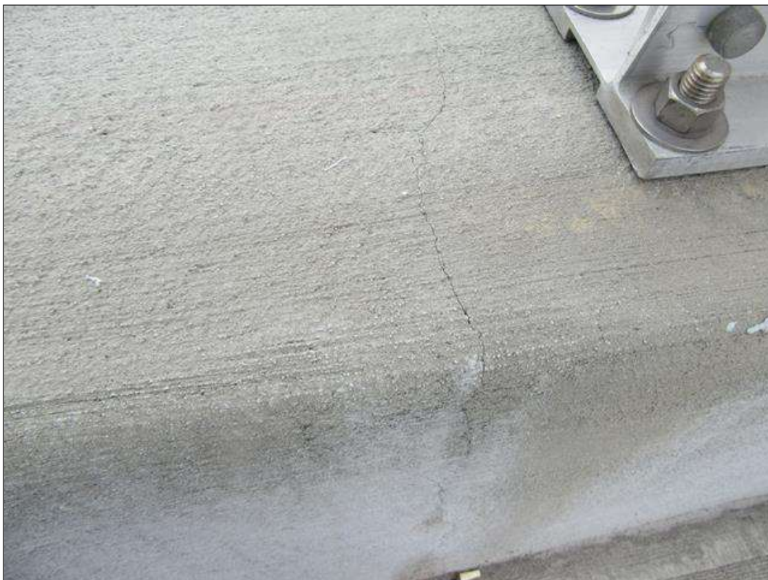
Span 2 Right Bridge Rail: HAIRLINE TRANSVERSE AND VERTICAL CRACKS AT 8- 10 FT. SPACING
