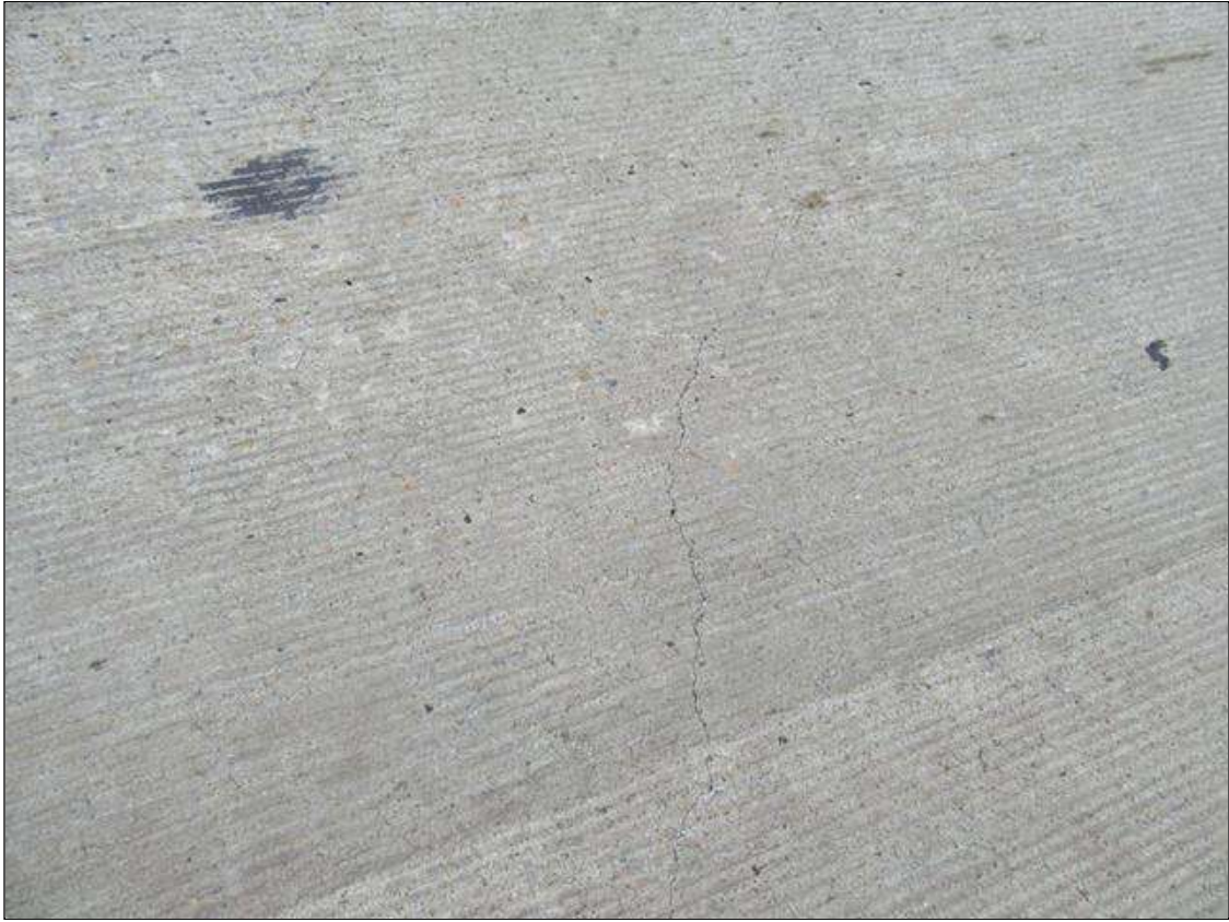
Approach 2: HAIRLINE LONGITUDINAL AND MAPCRACKING
