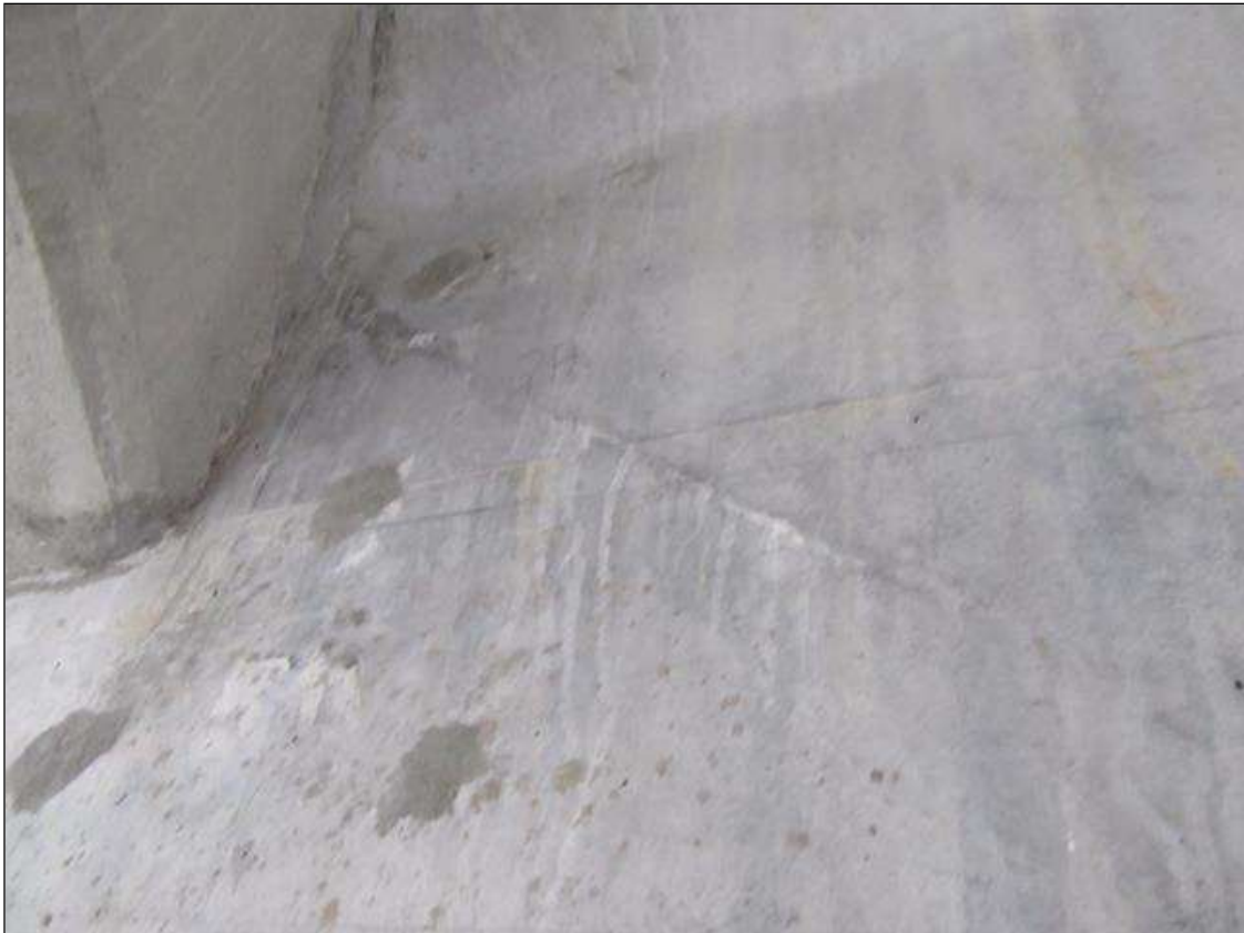
Span 2 Beam 4: 1 - 2 ' LONG X HAIRLINE DIAGONAL SHEER CRACKING IN WEB BAY 3 SIDE AT FAR END
