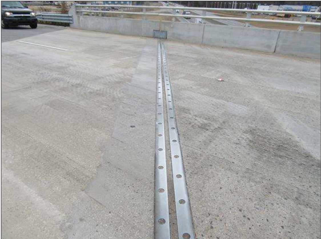
Expansion Joint : DEBRIS IN JOINT
