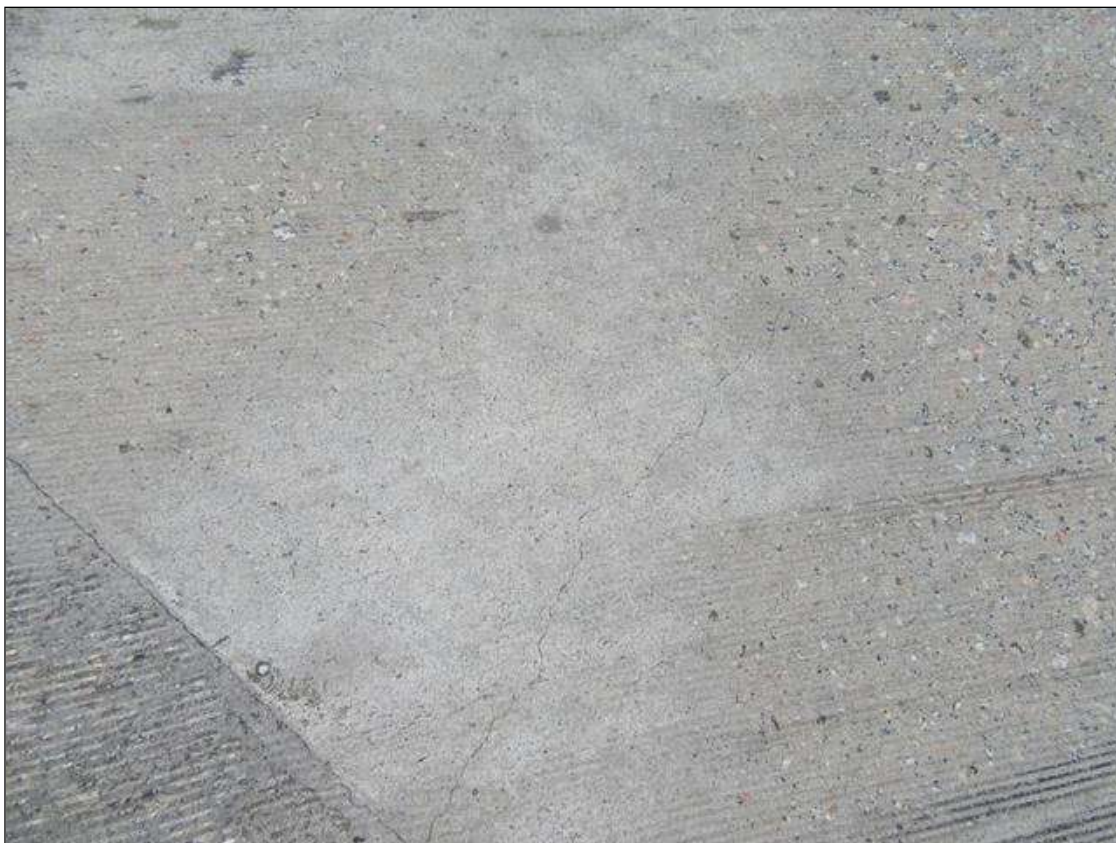
Span 1 Deck: HAIRLINE LONGITUDINAL CRACKING AT END BENT 1 END
