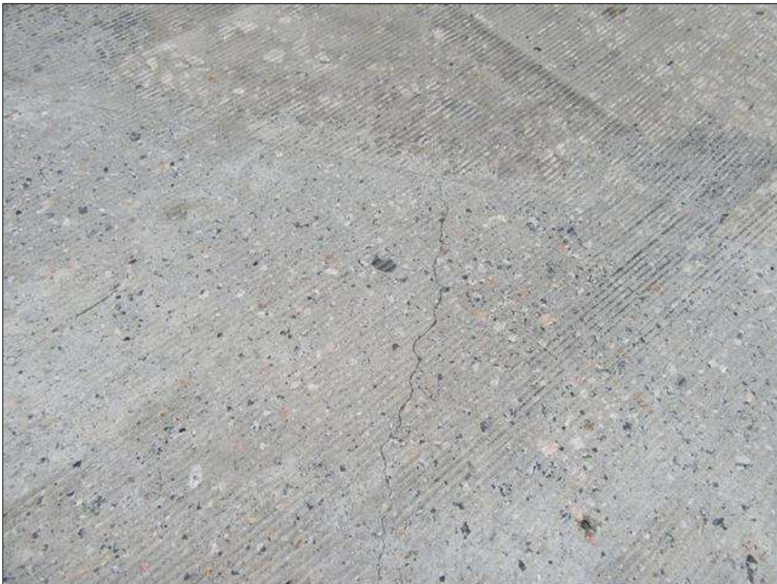
Approach 1: HAIRLINE LONGITUDINAL AND MAP CRACKING
