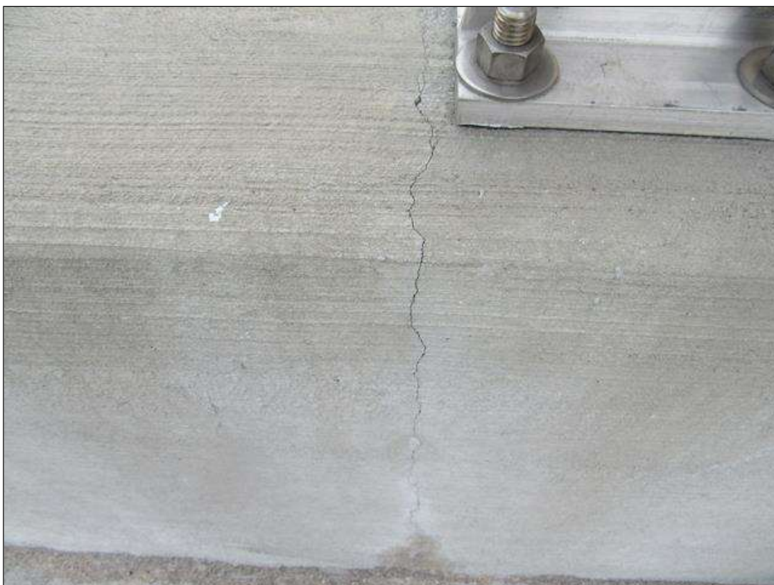
Span 2 Left Bridge Rail: HAIRLINE TRANSVERSE AND VERTICAL CRACKS AT 8- 10 FT. SPACING
