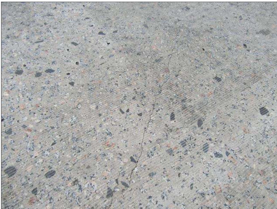
Span 2 Deck: HAIRLINE LONGITUDINAL CRACKING AT END BENT 2 END
