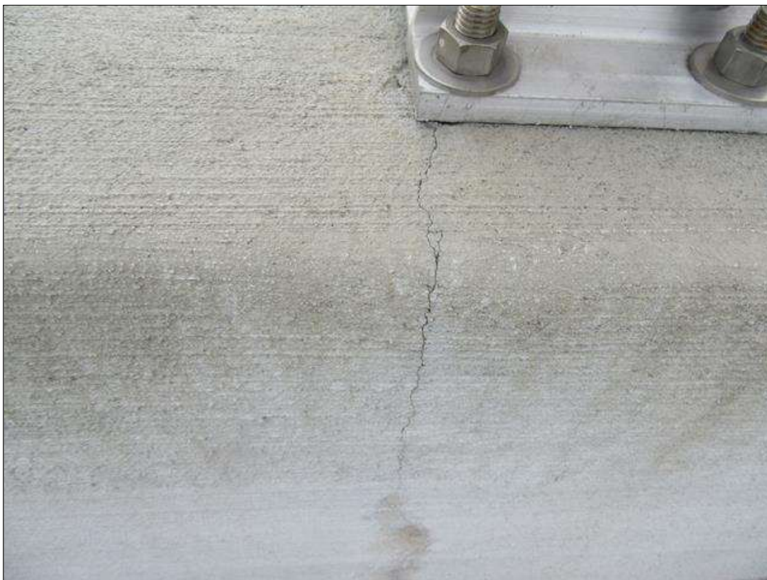
Span 1 Right Bridge Rail: HAIRLINE TRANSVERSE AND VERTICAL CRACK AT MID SPAN
