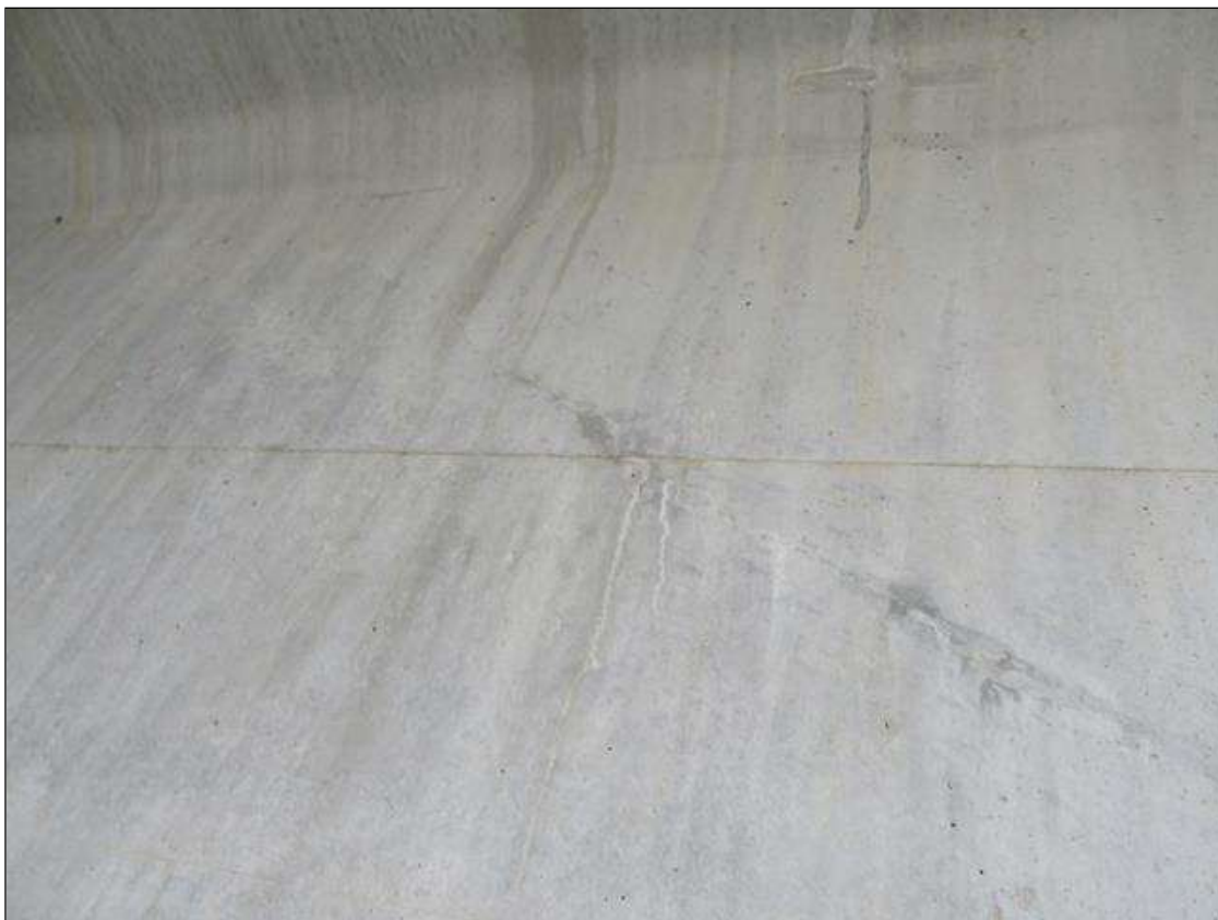
Span 2 Beam 1: 1- 2 ' LONG X HAIRLINE DIAGONAL SHEER CRACKING IN WEB LEFT SIDE AT FAR END
