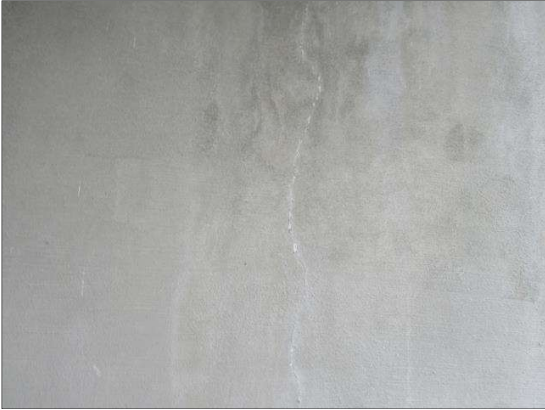
End Bent 1 Abutment/Backwall : 4' HIGH X HAIRLINE VERTICAL CRACK AT WEST END NEAR BEAM 1
