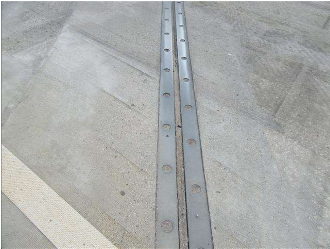
Expansion Joint : DEBRIS IN JOINT
