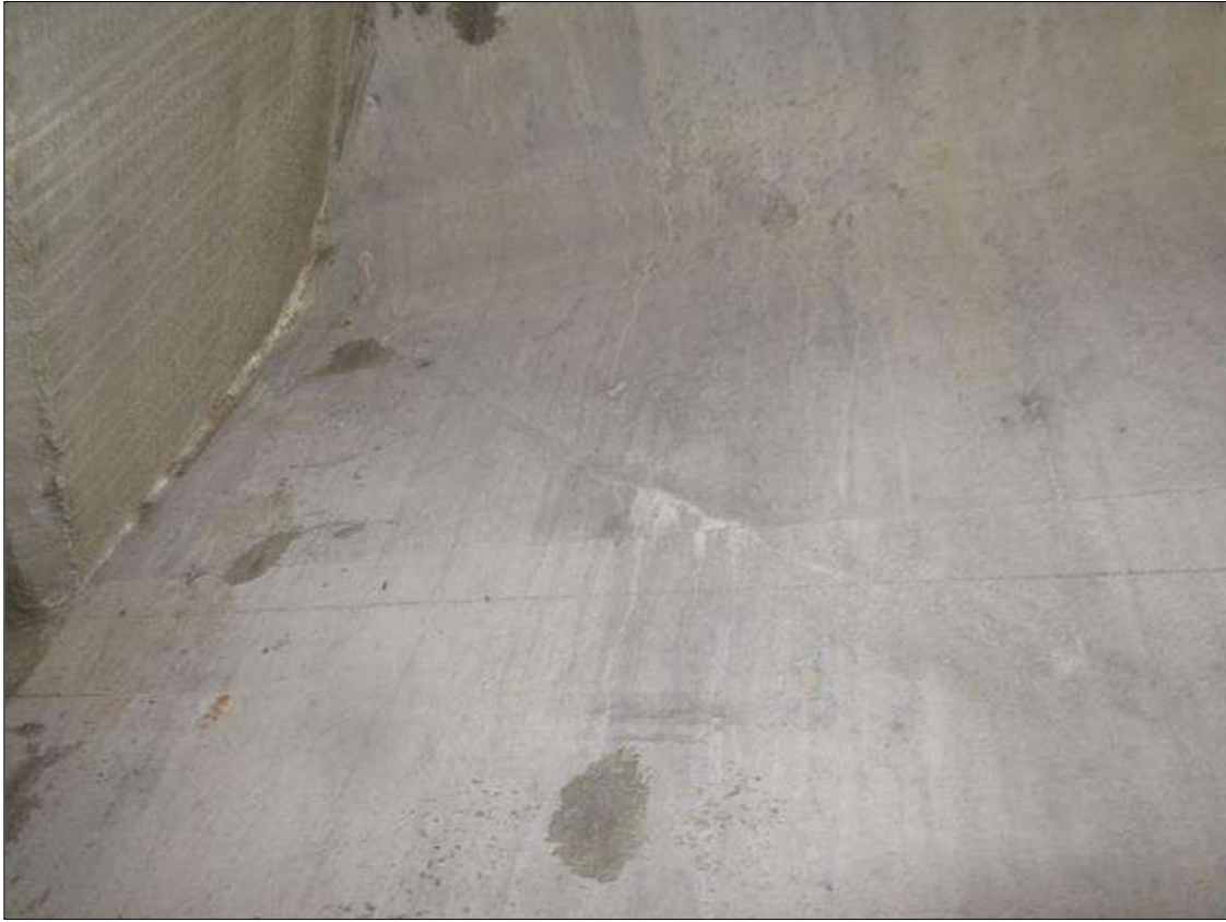
Span 2 Beam 3: 1- 2 ' LONG X HAIRLINE DIAGONAL SHEER CRACKING IN WEB BAY 2 SIDE AT FAR END
