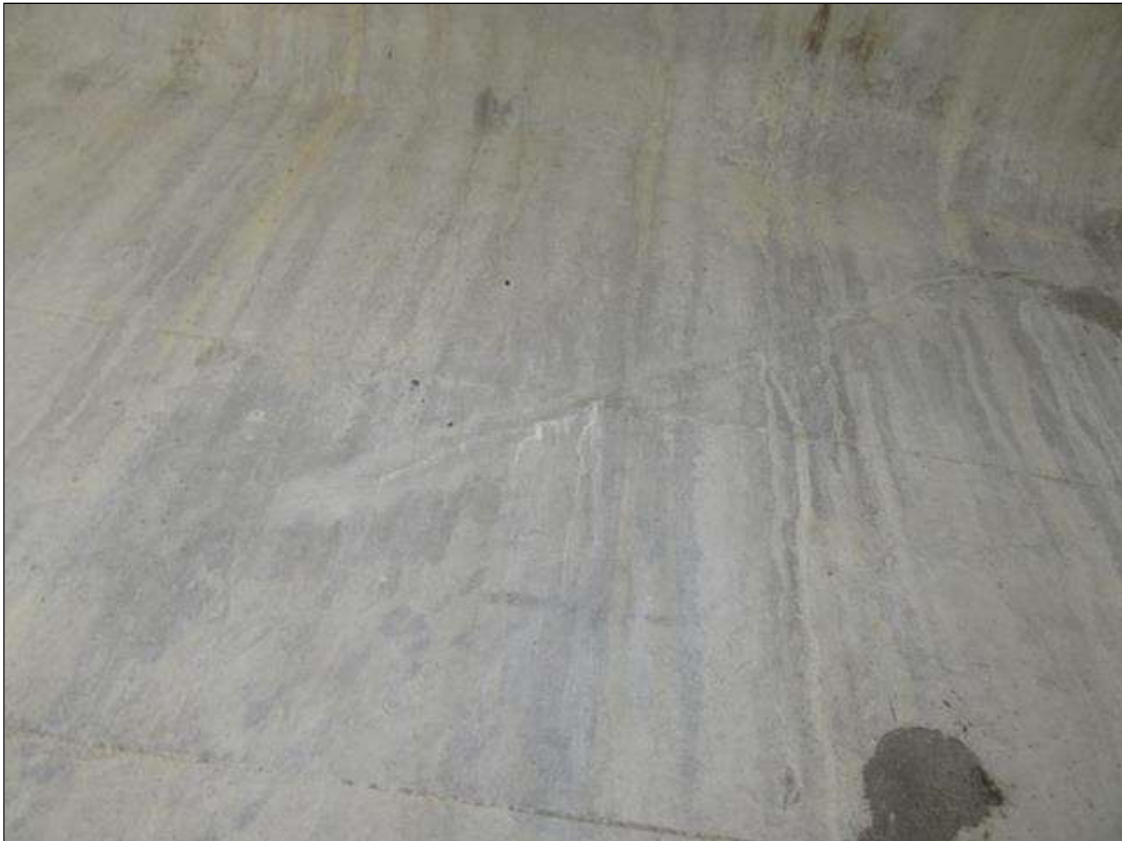
Span 2 Beam 2: 1- 2 ' LONG X HAIRLINE DIAGONAL SHEER CRACKING IN WEB BAY 2 SIDE AT FAR END
