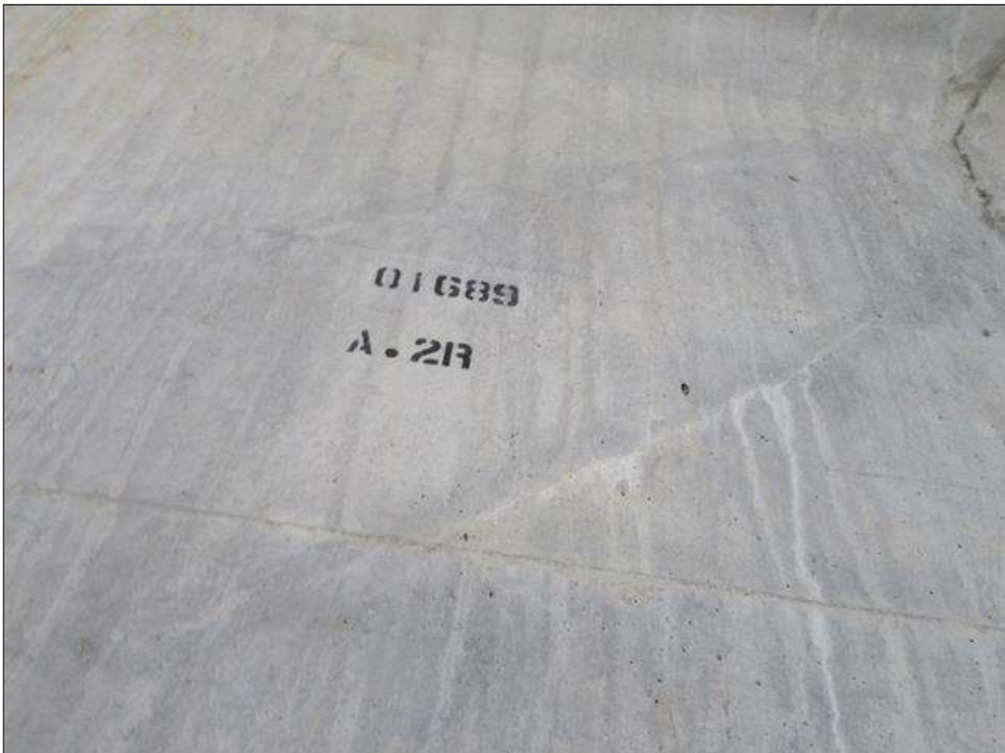
Span 1 Beam 2: 2 - 2' LONG X HAIRLINE DIAGONAL SHEER CRACKING IN WEB BAY 1 SIDE AT NEAR END
