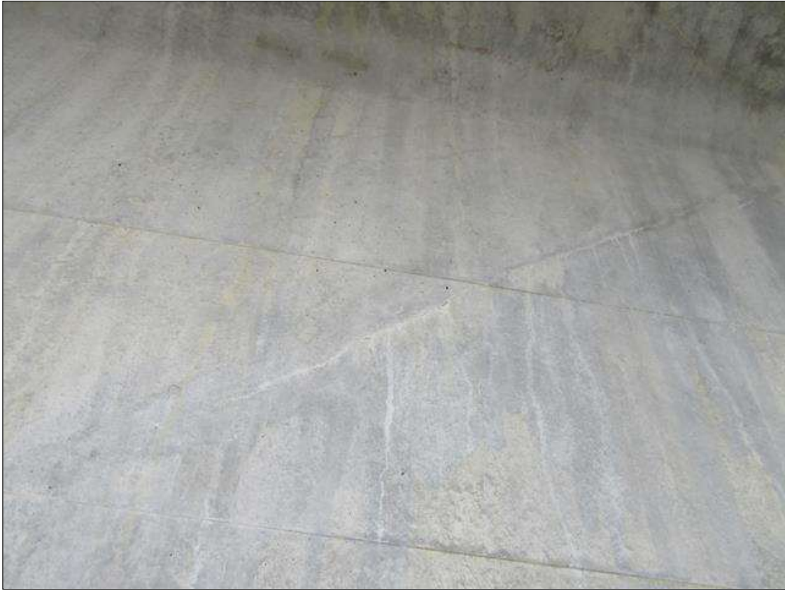
Span 2 Beam 4: 1 - 2 ' LONG X HAIRLINE DIAGONAL SHEER CRACKING IN WEB RIGHT SIDE AT FAR END
