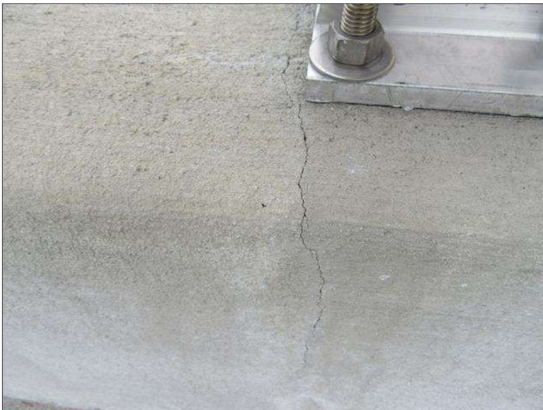
Span 1 Left Bridge Rail: HAIRLINE TRANSVERSE AND VERTICAL CRACKS AT 8- 10 FT. SPACING
