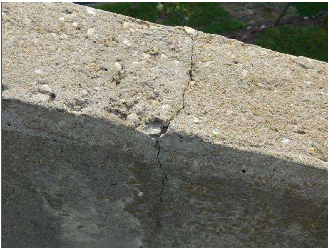
Span 3 Right Bridge Rail: HAIRLINE TRANSVERSE AND VERTICAL CRACKS AT 1-4 FT. SPACING
