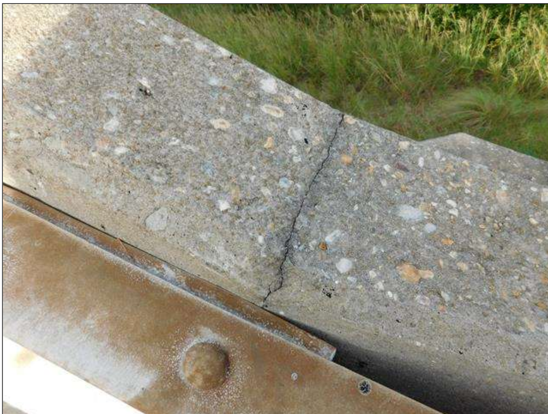
Span 4 Left Bridge Rail: HAIRLINE TRANSVERSE AND VERTICAL CRACKING
