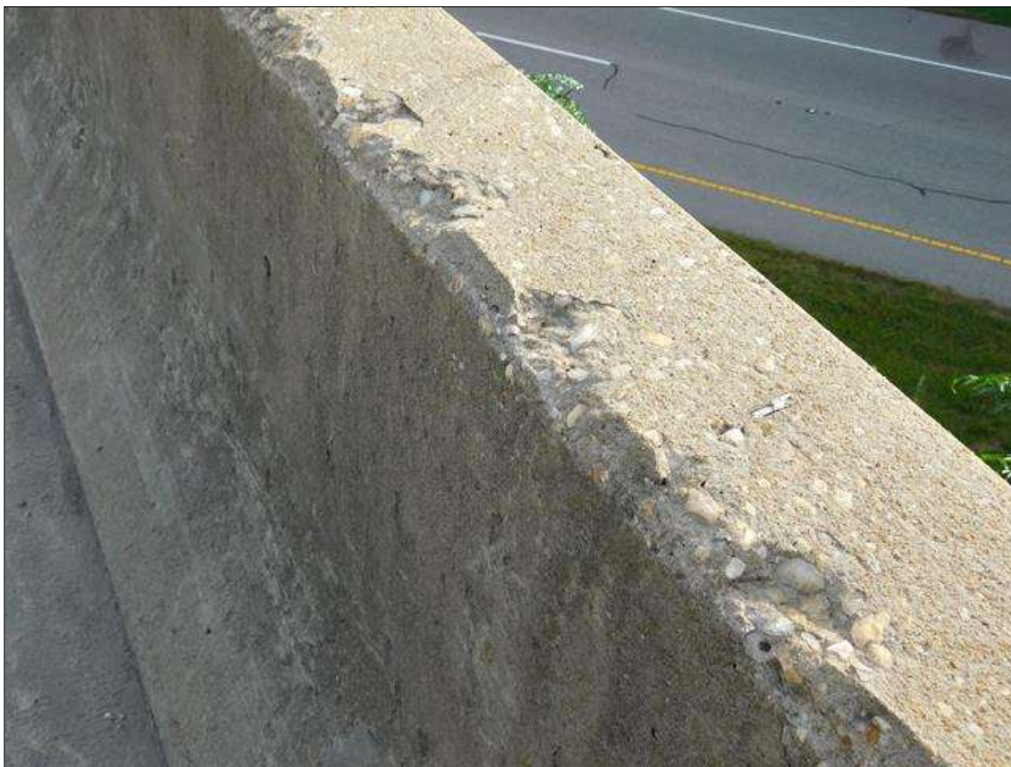
Span 1 Right Bridge Rail: SURFACE SPALL 4 FT. LONG X 2" WIDE X 1" DEEP IN TOP OF RAIL AT 20 FT. FROM END BENT 1
