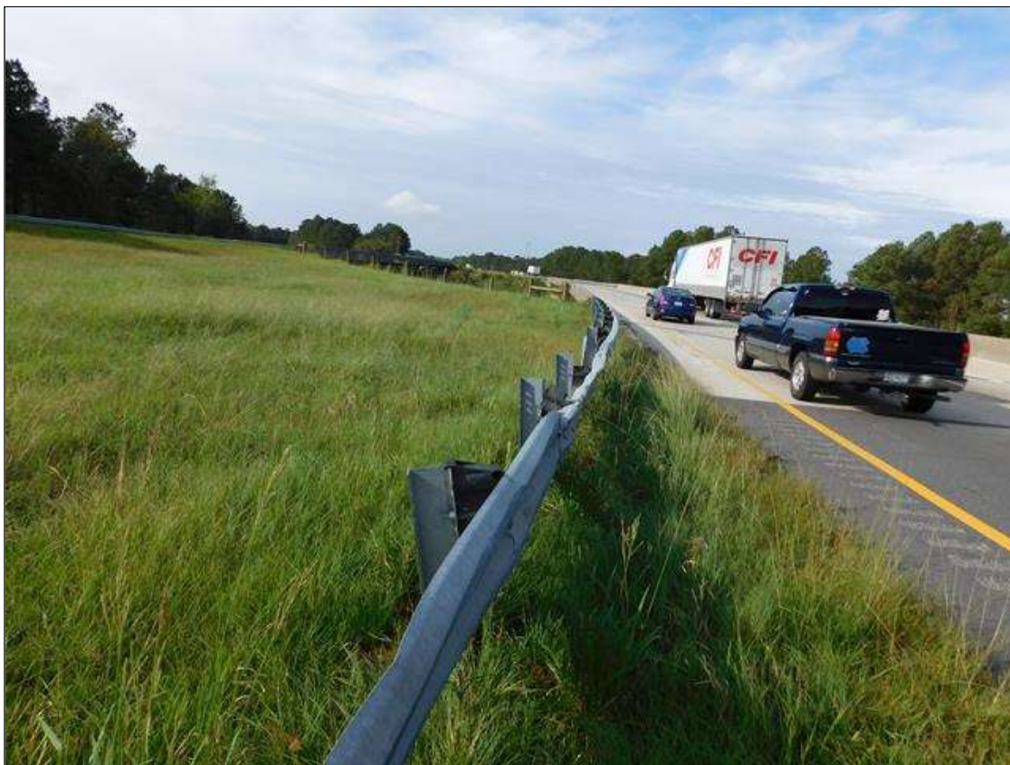
20 FT. GUARDRAIL AND 4 POSTS DAMAGED AT NORTHEAST CORNER
