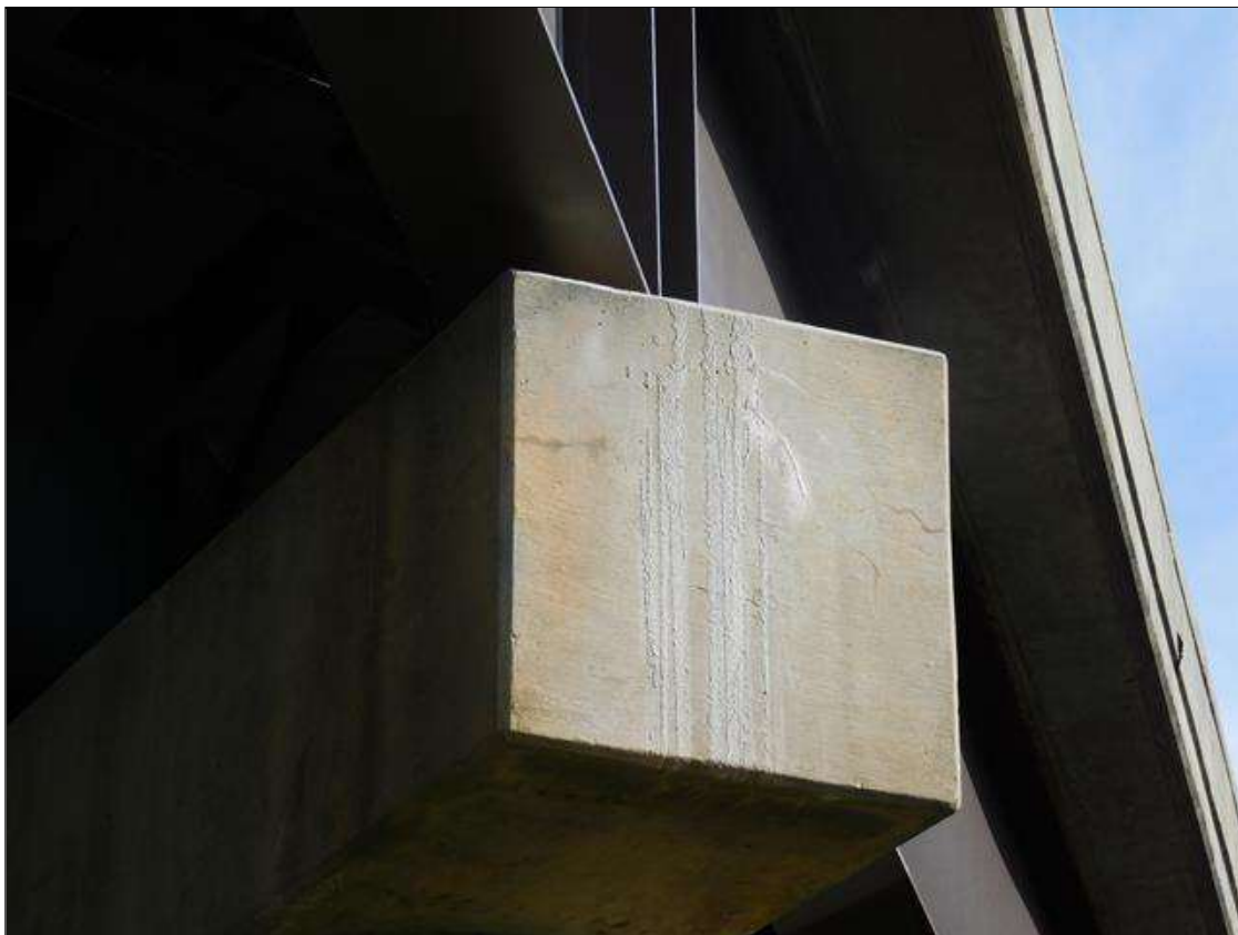
Bent 2 Cap 1: HAIRLINE MAP CRACKING WITH EFFLO ON EAST END OF CAP
