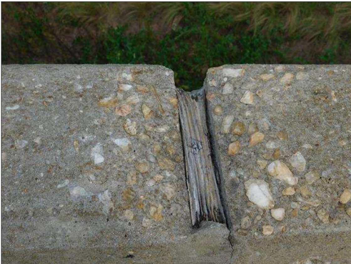
Span 1 Left Bridge Rail: SPALL 6" LONG X 2" WIDE X 1 1/2" DEEP IN TOP OF RAIL AT MID SPAN
