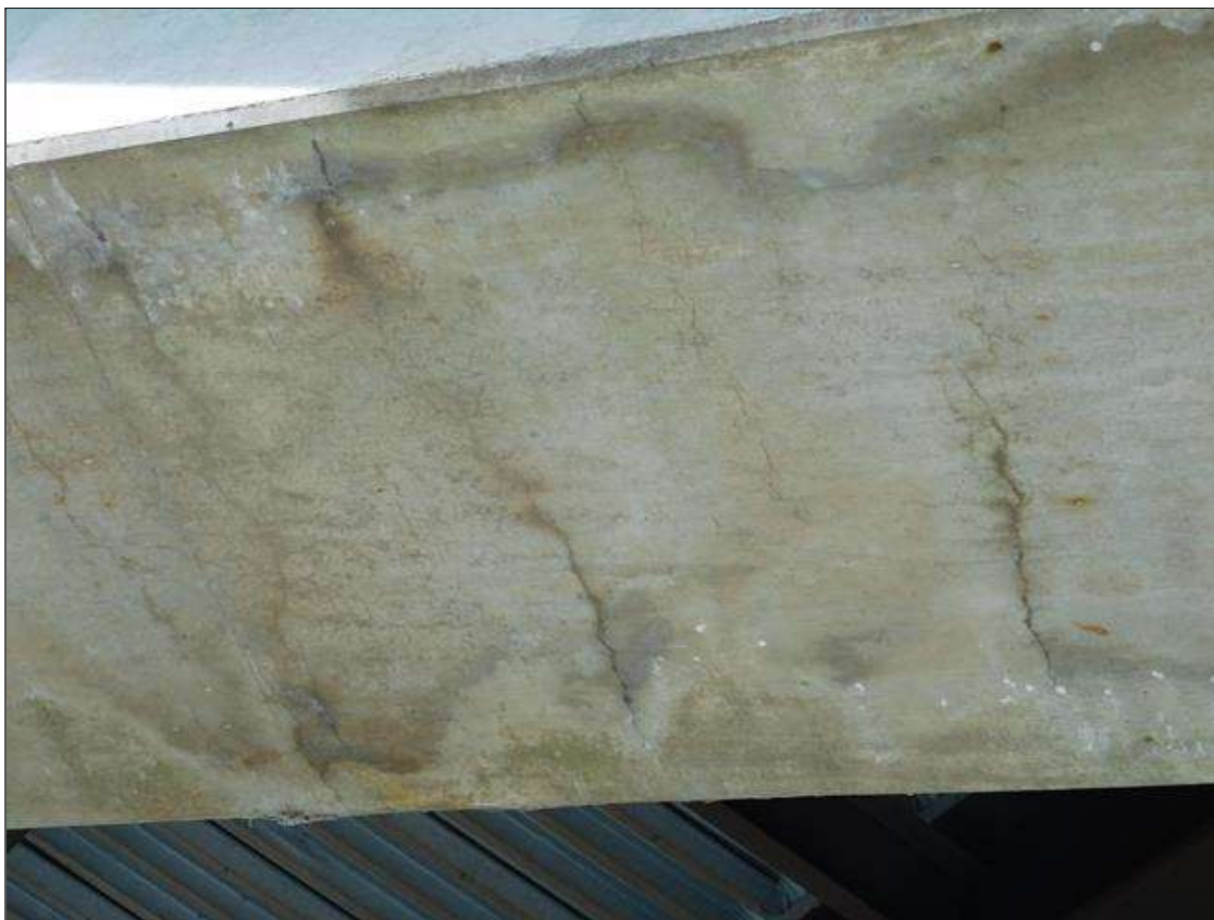
Bent 1 Cap 1: 3 - 3 FT. LONG X HAIRLINE TRANSVERSE CRACKS AT 2 FT. SPACING IN BOTTOM OF CAP BETWEEN COLUMNS 3 AND 4
