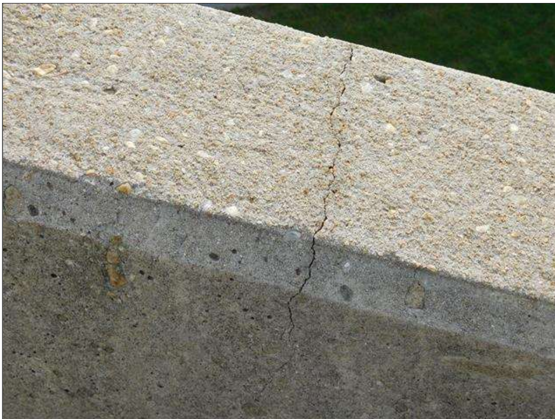
Span 1 Right Bridge Rail: HAIRLINE TRANSVERSE AND VERTICAL CRACKS AT 1-4 FT. SPACING
