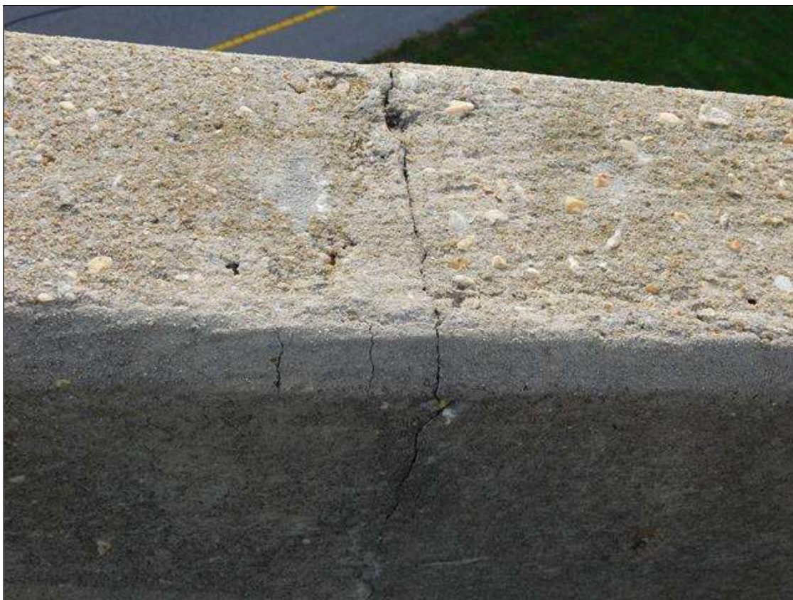
Span 2 Right Bridge Rail: HAIRLINE TRANSVERSE AND VERTICAL CRACKS AT 1-4 FT. SPACING
