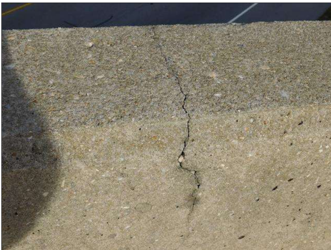
Span 2 Left Bridge Rail: HAIRLINE TRANSVERSE AND VERTICAL CRACKING
