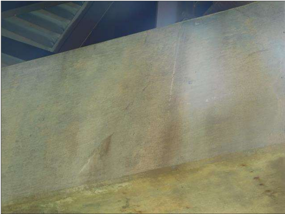
Bent 2 Cap 1: 1/32" WIDE DIAGONAL CRACK IN SPAN 2 FACE OF CAP EAST END UNDER BEAM 6
