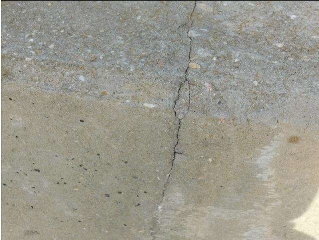
Span 1 Left Bridge Rail: HAIRLINE TRANSVERSE AND VERTICAL CRACKING
