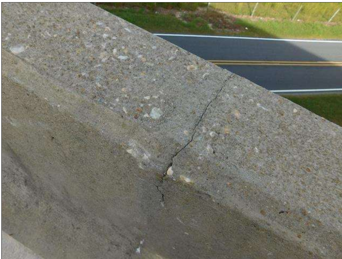
Span 3 Left Bridge Rail: HAIRLINE TRANSVERSE AND VERTICAL CRACKING
