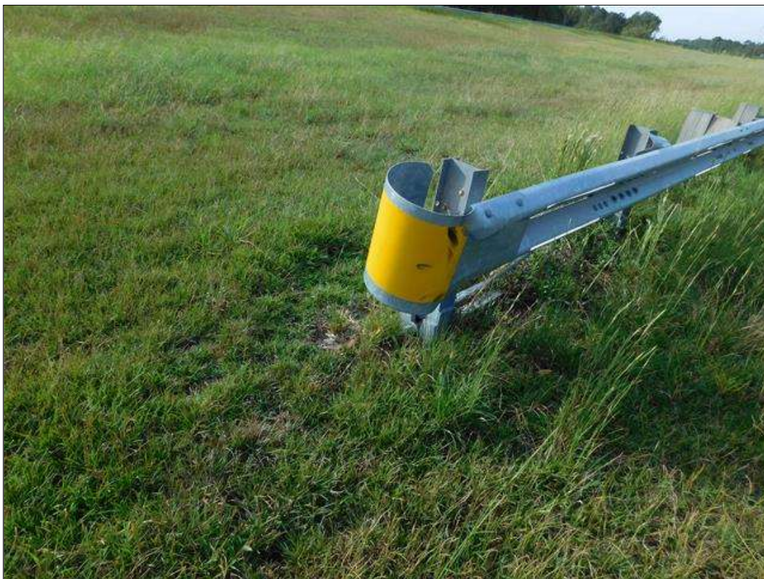
GUARDRAIL END TERMINAL
