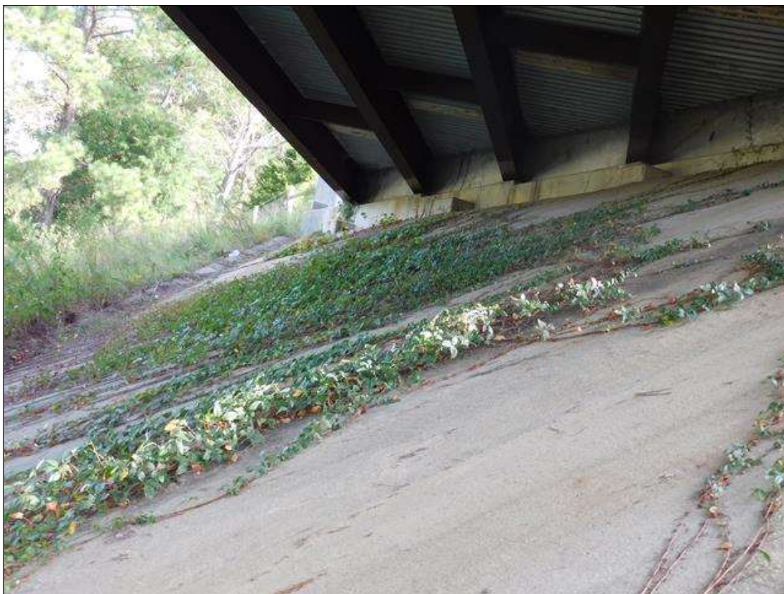
VEGETATION ON END BENT 2 SLOPE 100 FT
