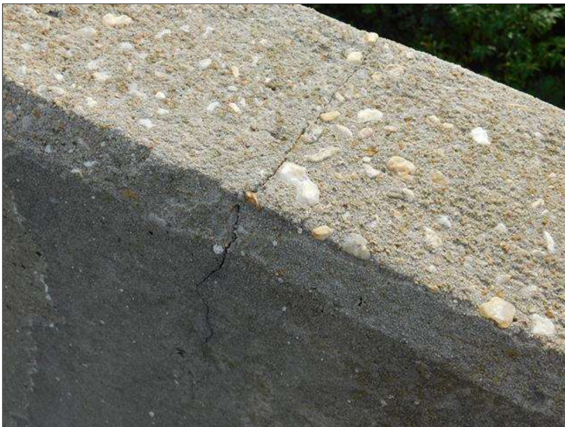
Span 4 Right Bridge Rail: HAIRLINE TRANSVERSE AND VERTICAL CRACKS AT 1-4 FT. SPACING
