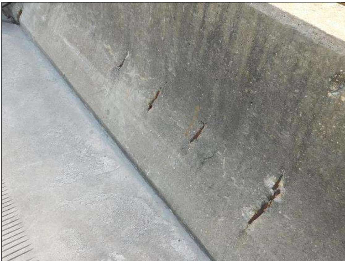
Span 4 Right Bridge Rail: 4 - 2" HIGH X 1/2" DEEP SURFACE SPALLS WITH EXPOSED REBAR NEAR END BENT 2
