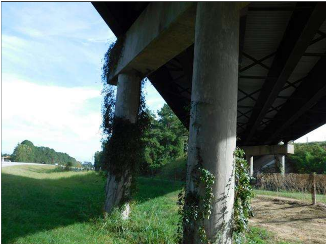
VEGETATION ON ALL COLUMNS AT BENT 2
