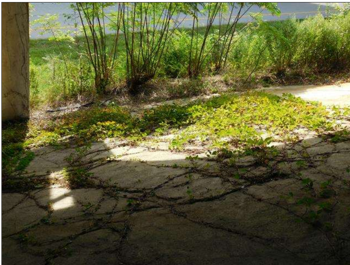
50 SQUARE FOOT. FT. VEGETATION ON END BENT 1 SLOPE
