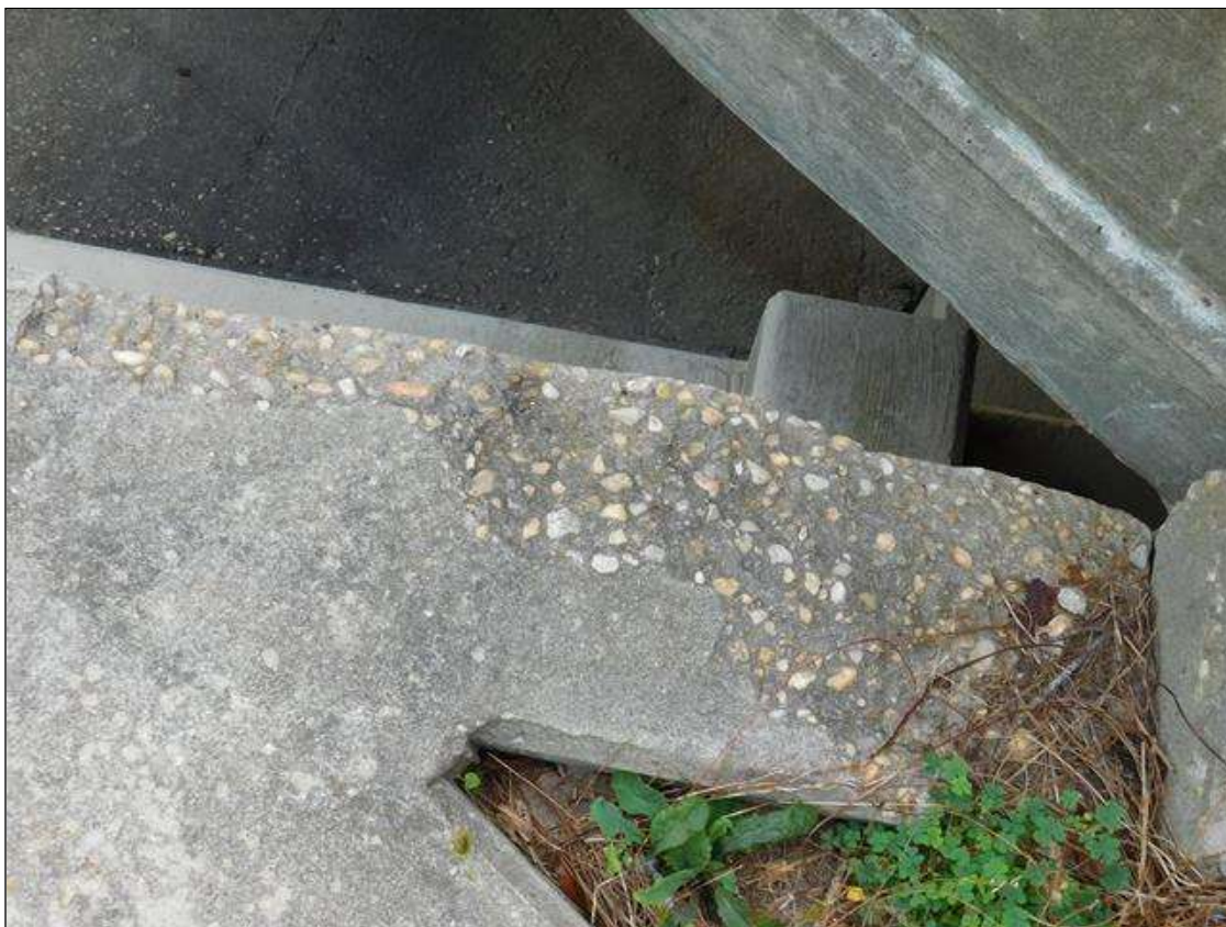
SOUTHWEST WINGWALL TOP SPALLED 4 FT. LONG X 12" WIDE X UP TO 4" DEEP
