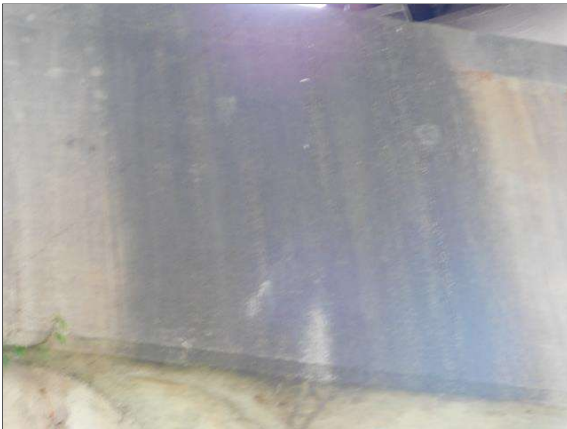
Bent 2 Cap 1: 1/32" WIDE DIAGONAL CRACK ON SPAN 2 FACE UNDER BEAM 6
