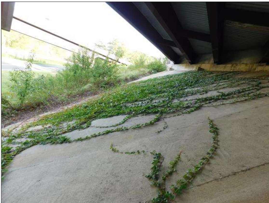
VEGETATION ON END BENT 2 SLOPE PROTECTION 100 SQUARE FOOT. FT.
