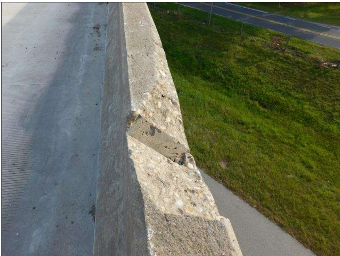
Span 2 Right Bridge Rail: SPALL 42" LONG X 7" WIDE X 6" DEEP AT MID SPAN PRIORITY MAINTENANCE ISSUED
