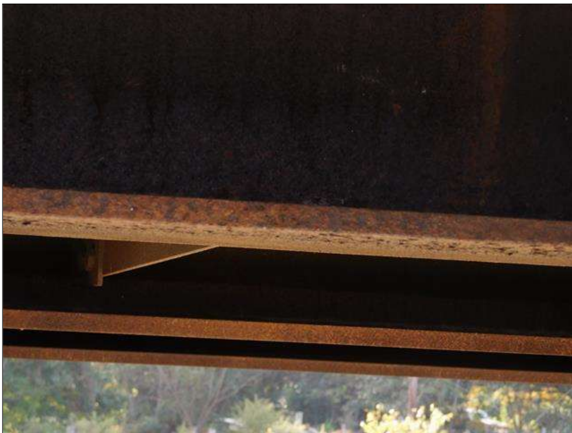
SPAN 2 BEAM 4 AT 10 FT. FROM BENT 1 SIDE VIEW OF SURFACE RUST ON BOTTOM FLANGE, NO SECTION LOSS
