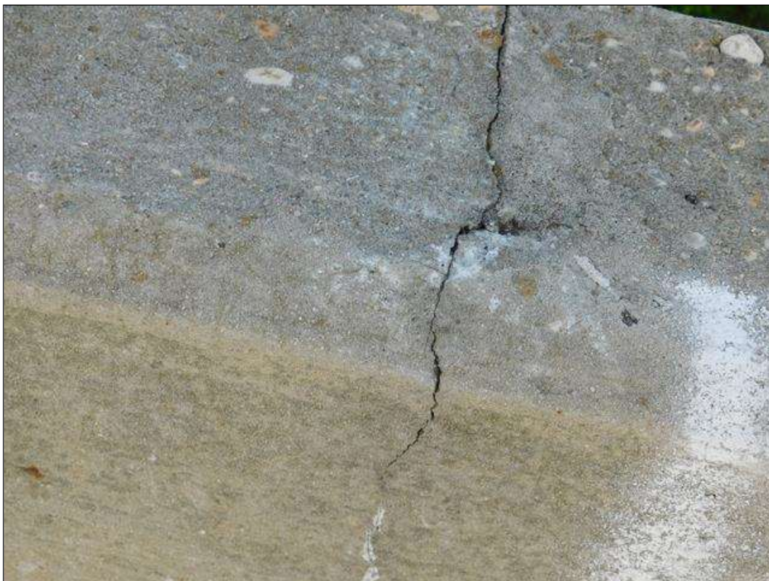
Span 2 Right Bridge Rail: HAIRLINE TRANSVERSE AND VERTICAL CRACKS AT 1-3 FT. SPACING
