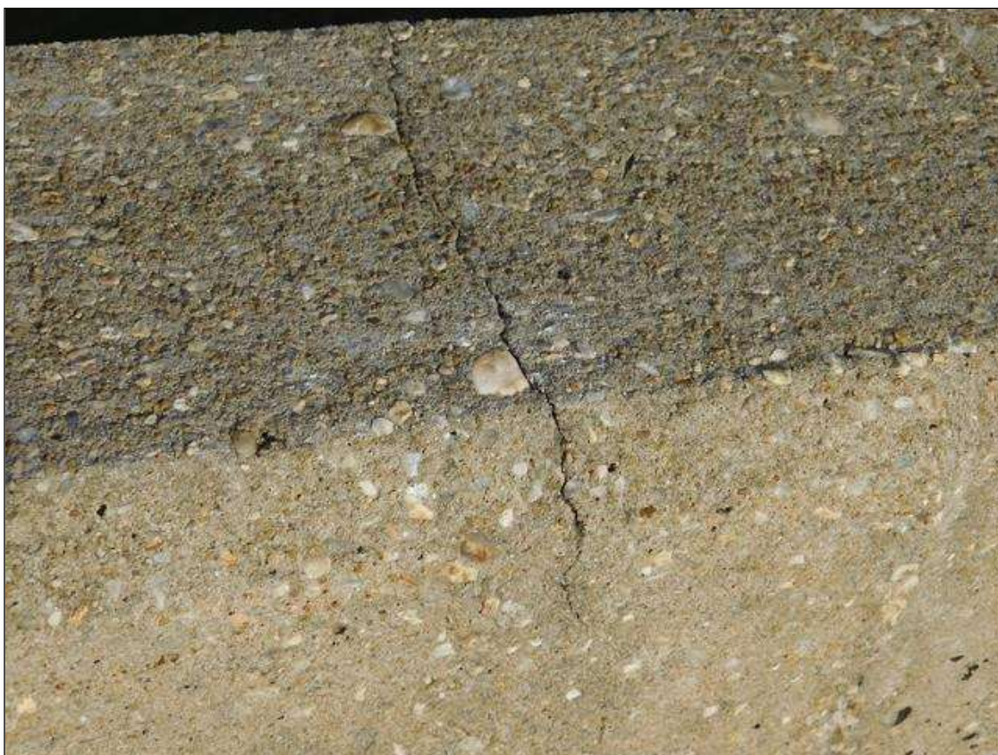
Span 3 Left Bridge Rail: HAIRLINE TRANSVERSE AND VERTICAL CRACKS AT 1-3 FT. SPACING
