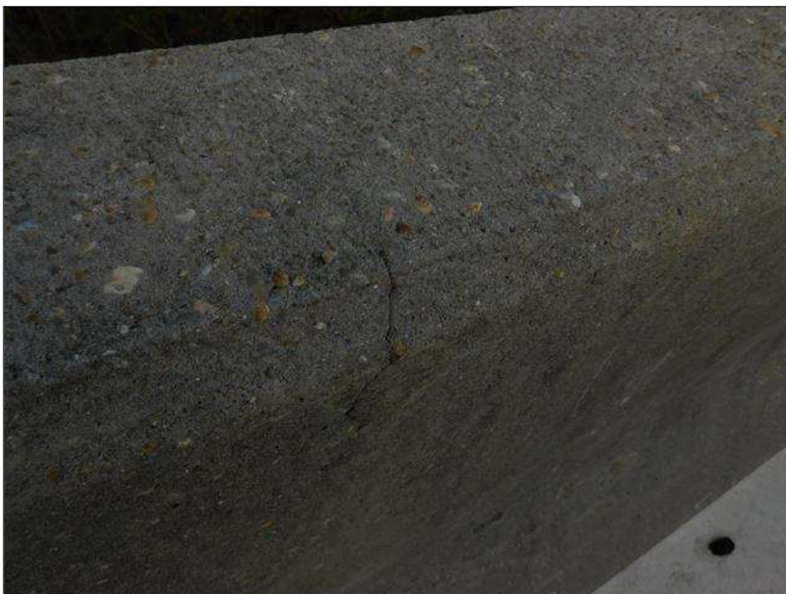
Span 1 Left Bridge Rail: HAIRLINE TRANSVERSE AND VERTICAL CRACKS AT 1-3 FT. SPACING
