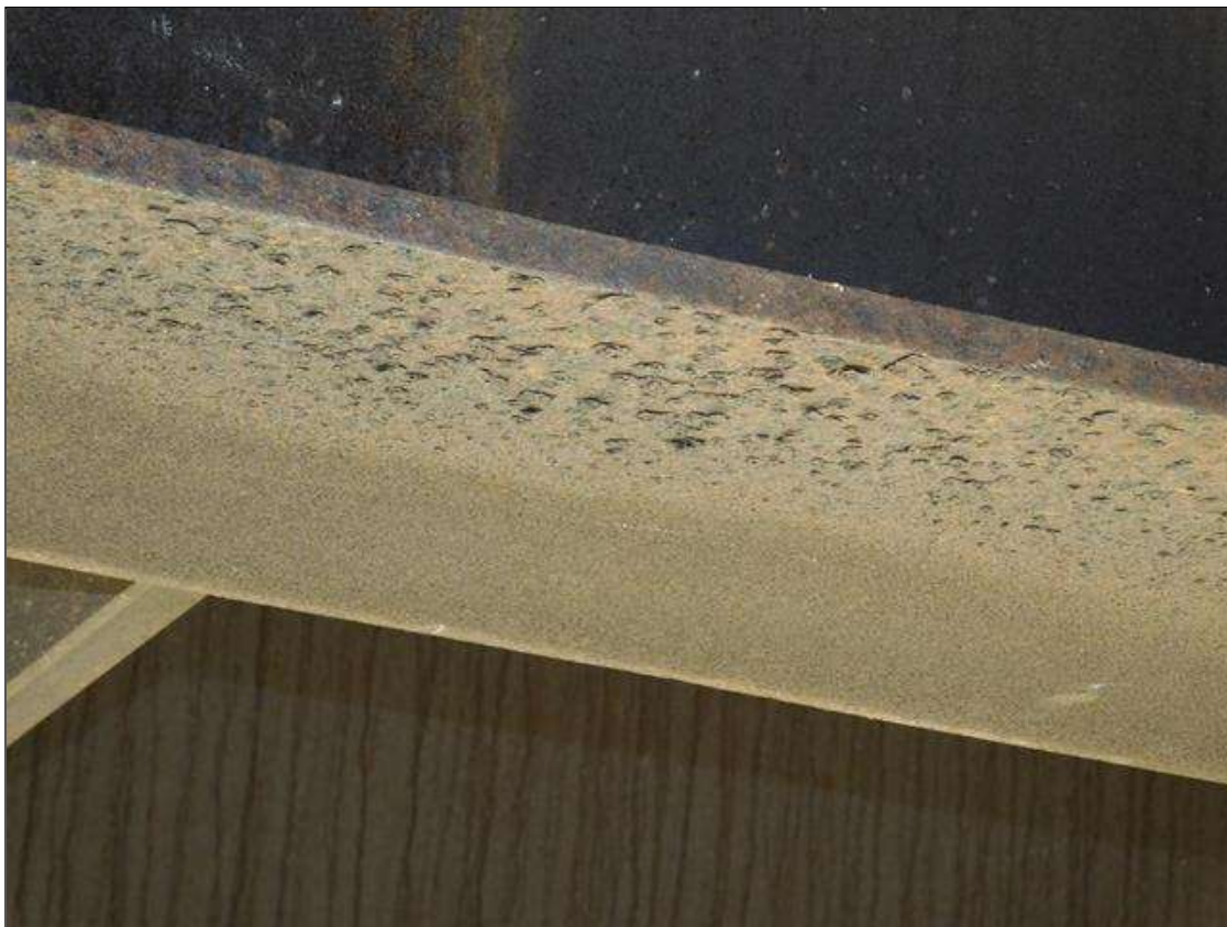
Span 2 Beam 4: SURFACE RUST ON BOTTOM FLANGE 10' LONG X 8" WIDE WITH NO SECTION LOSS AT 10' FROM BENT 1
