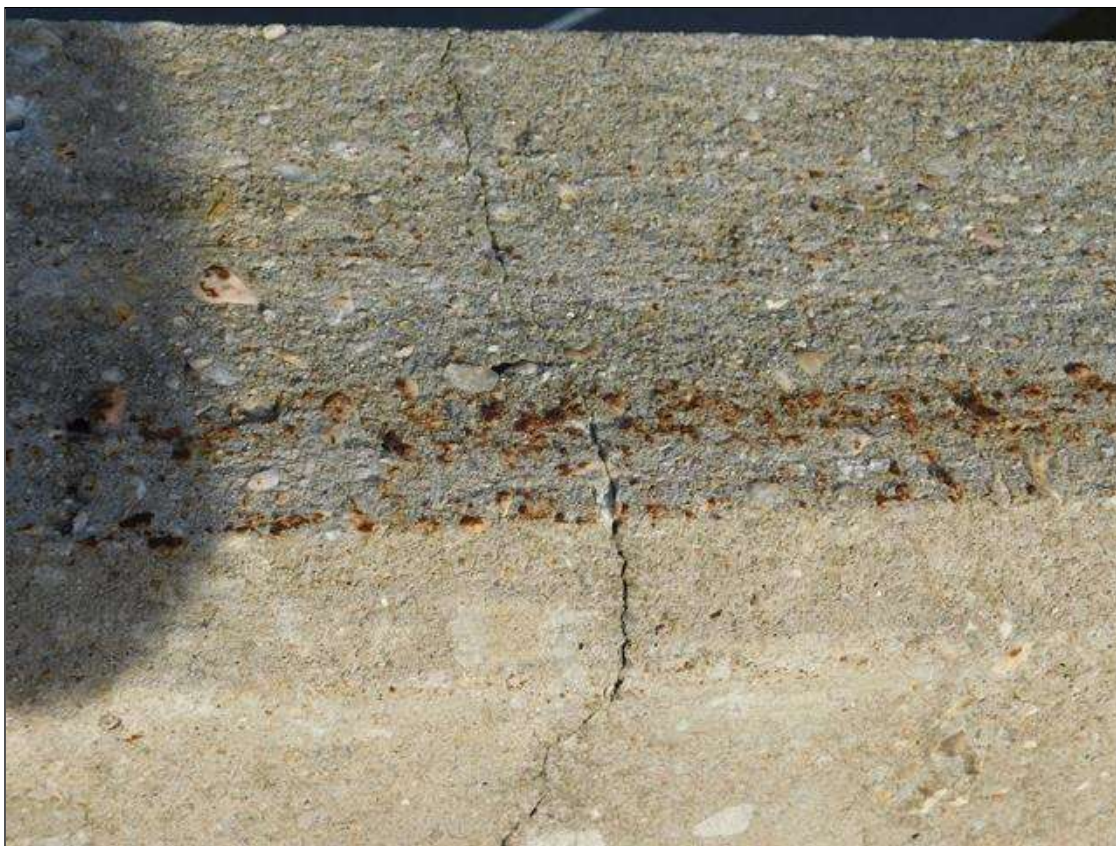
Span 2 Left Bridge Rail: HAIRLINE TRANSVERSE AND VERTICAL CRACKS AT 1-3 FT. SPACING
