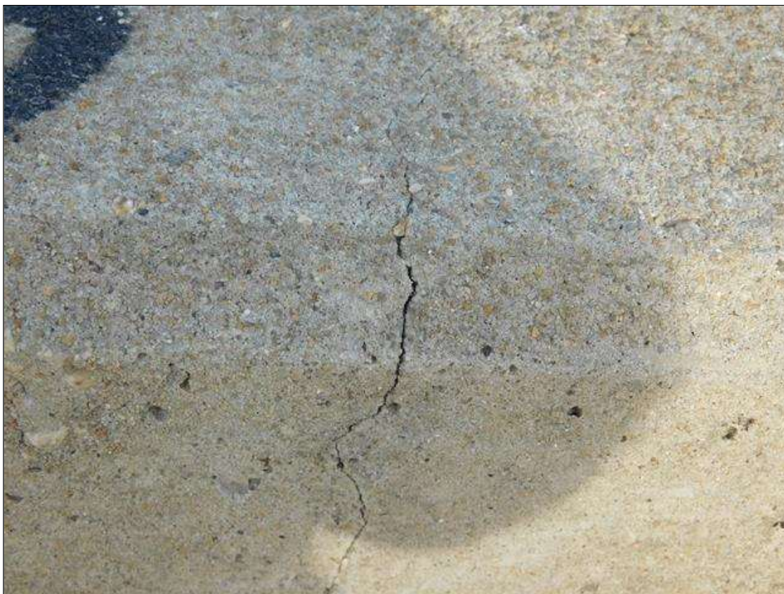
Span 4 Left Bridge Rail: HAIRLINE TRANSVERSE AND VERTICAL CRACKS AT 1-3 FT. SPACING
