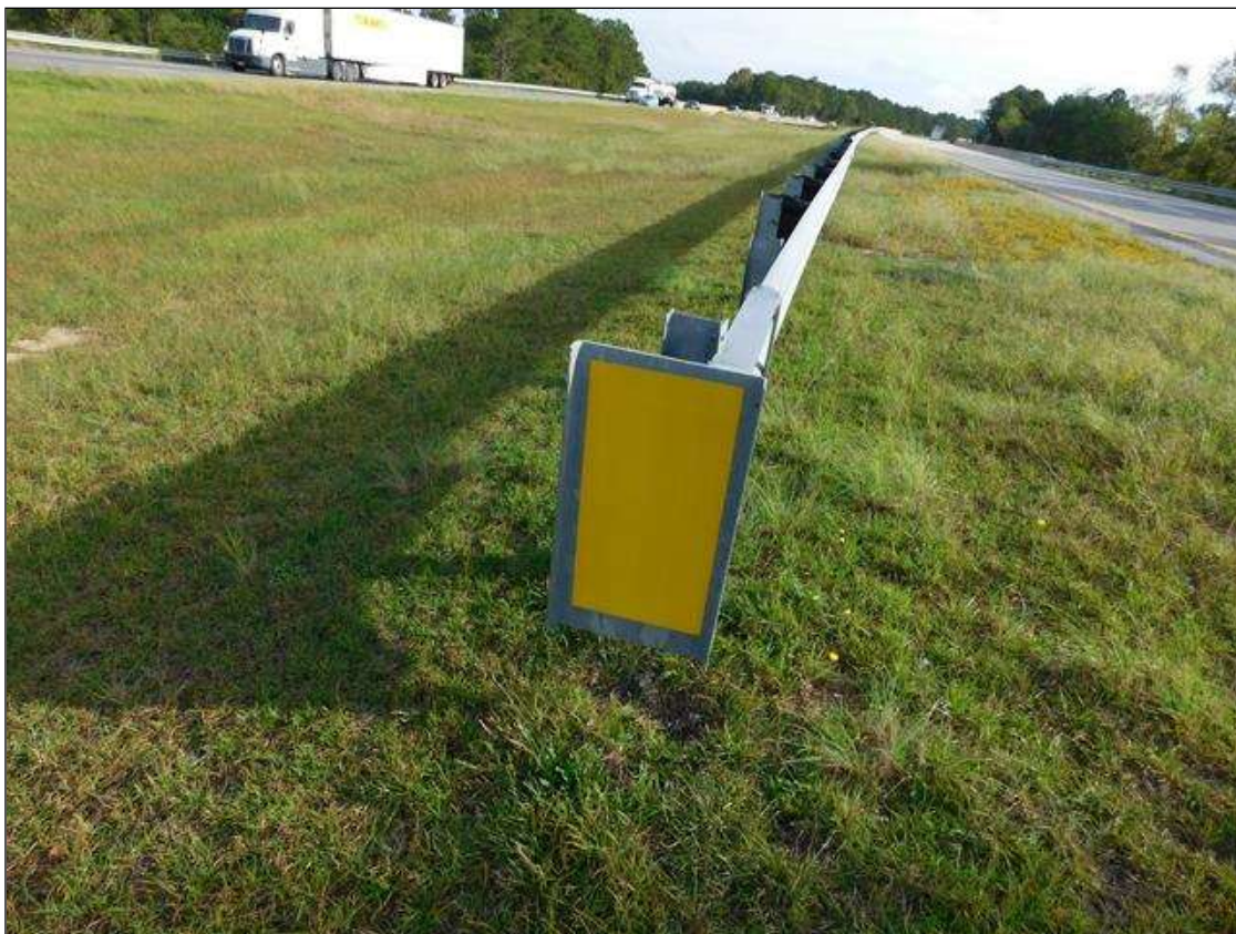
GUARDRAIL END TERMINAL
