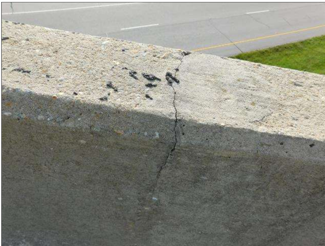
Span 1 Right Bridge Rail: HAIRLINE TRANSVERSE AND VERTICAL CRACKS AT 1-3 FT. SPACING
