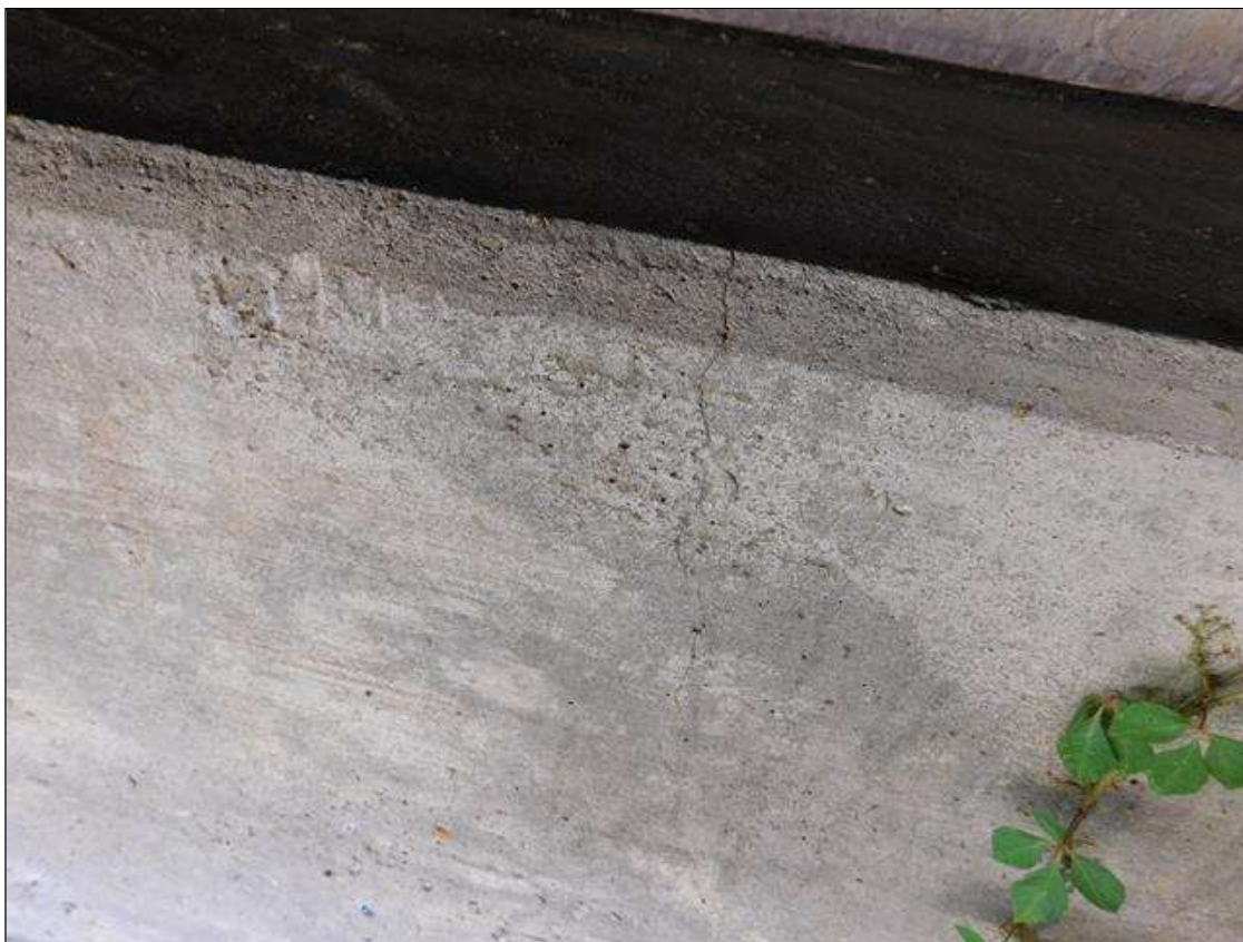
End Bent 2 Cap 1: 6 - HAIRLINE VERTICAL CRACKS AT 1' SPACING IN END BENT 2 CAP FROM BAY 1 TO BEAM 3
