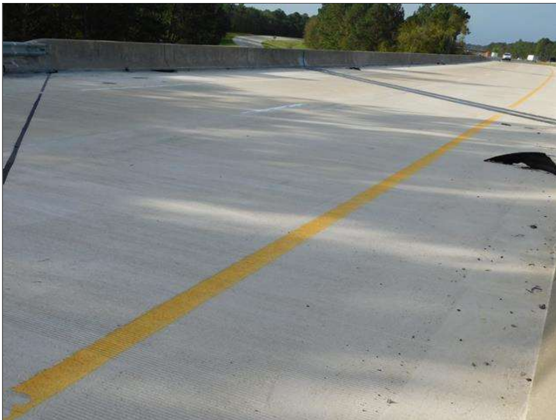
SPAN 4 DECK MILLED AND RESURFACED WITH SAME MEASUREMENTS, ALL SPANS ARE SIMILAR 2018
