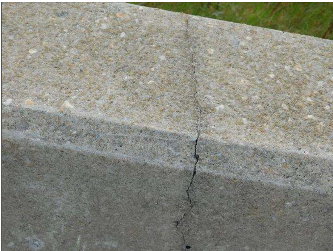
Span 4 Right Bridge Rail: HAIRLINE TRANSVERSE AND VERTICAL CRACKS AT 1-3 FT. SPACING
