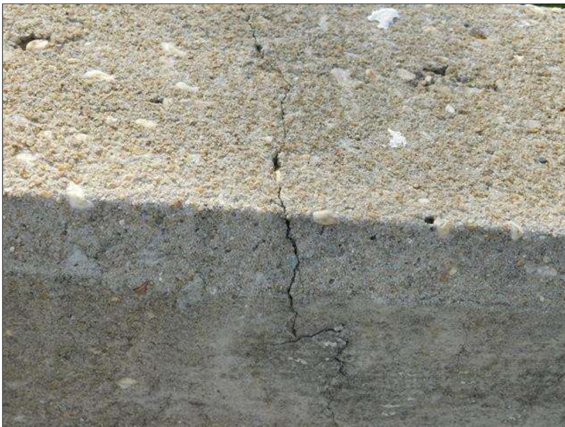
Span 3 Right Bridge Rail: HAIRLINE TRANSVERSE AND VERTICAL CRACKS AT 1-3 FT. SPACING
