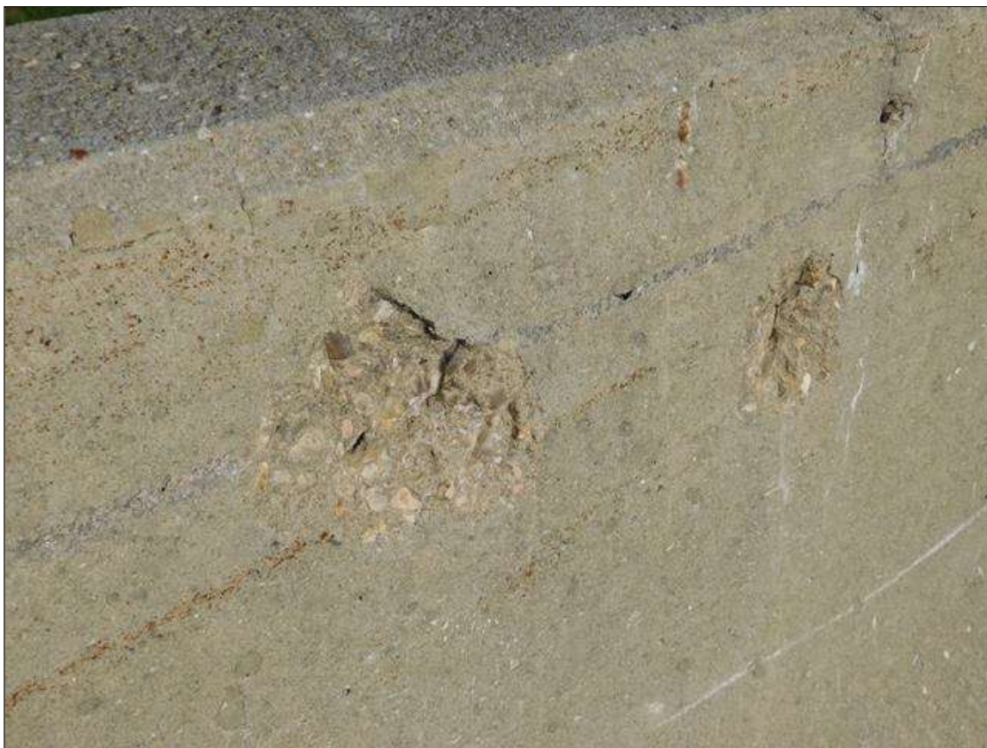
Span 2 Right Bridge Rail: 2 - 6" DIAMETER X 1" DEEP SURFACE SPALLS
