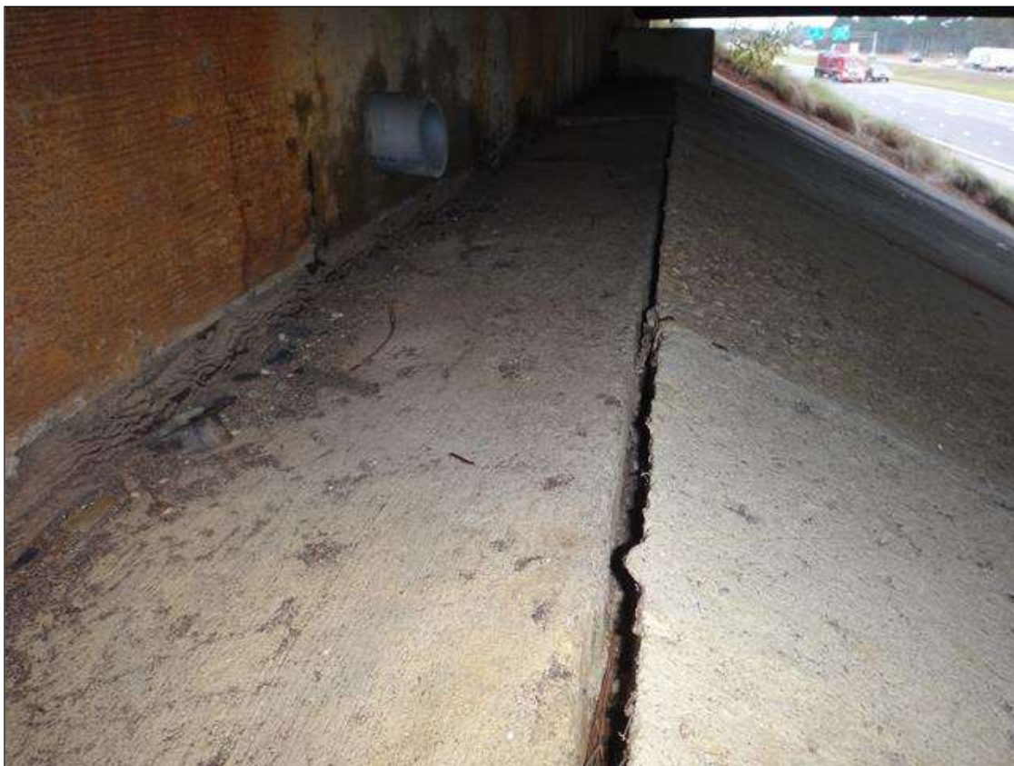
top face of slope protection below bay 5, seperated and settled (8ft x up to 3/4in x 5in) (photo 2 of 2)
