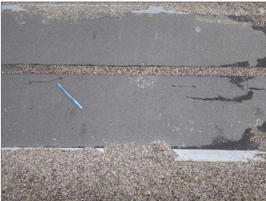
Expansion Joint 3: eastbound lane at 5ft from rail, (4) longitudinal cracks in header (up to 11in x up to 1/8in)
