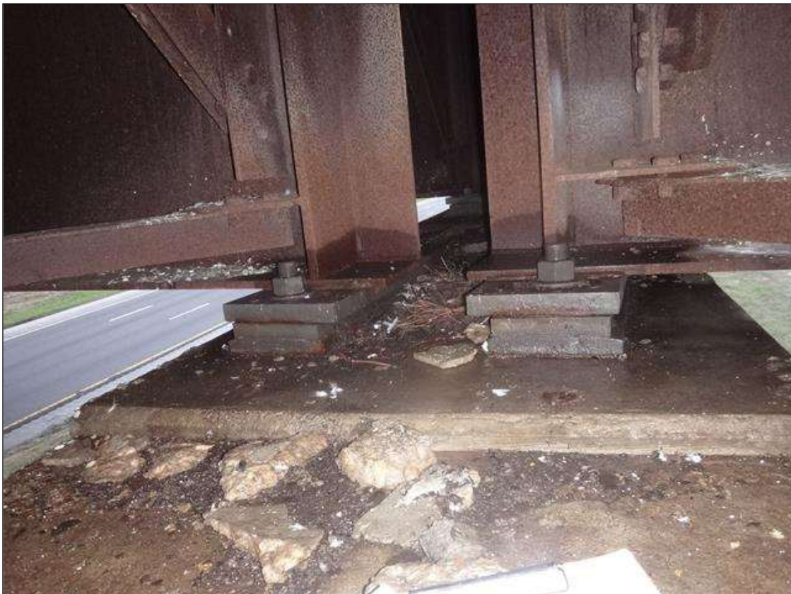
interior bearing assembly
