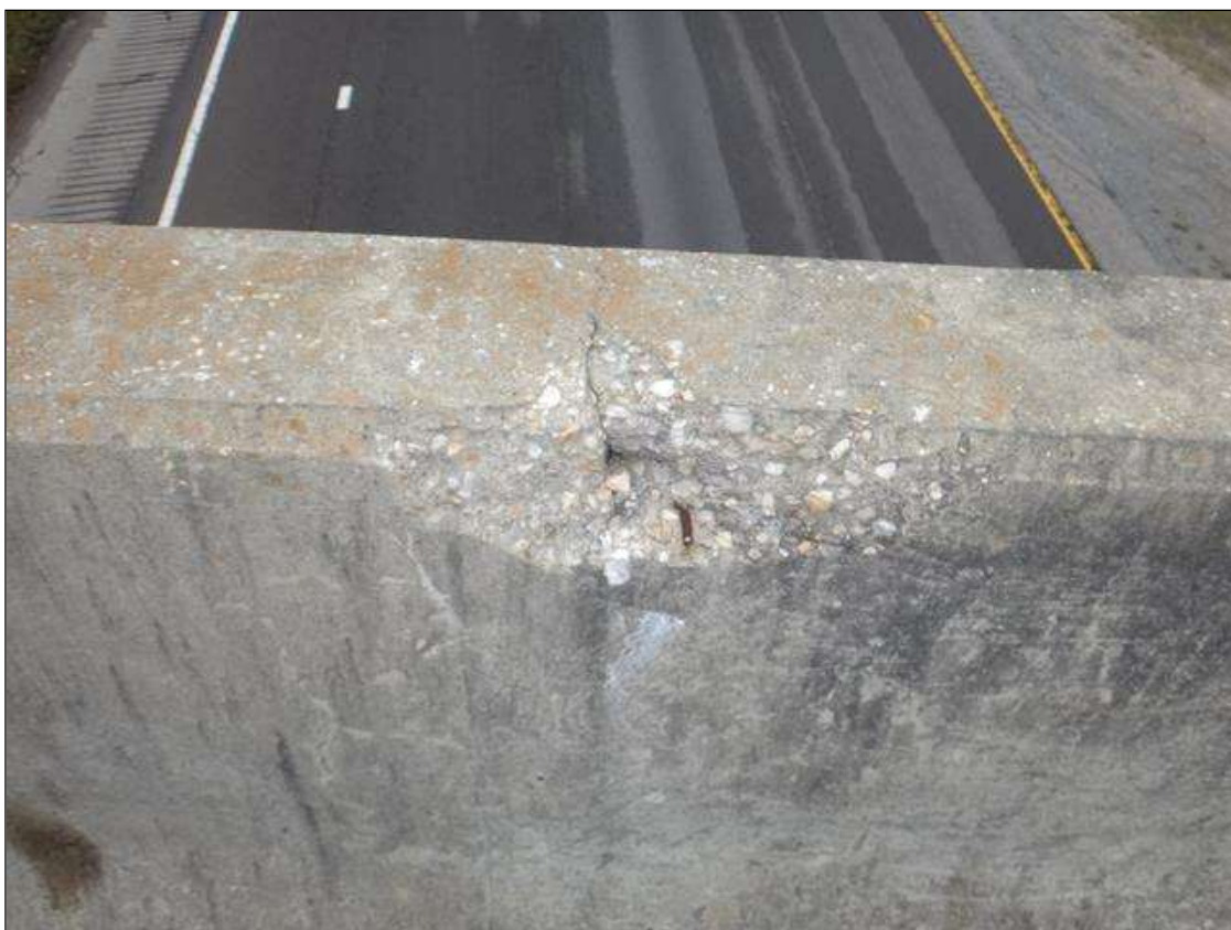
Span 1 Left Bridge Rail: top of rail at 60ft from end bent 1, spall (14in x 5in x 2-1/2in)
