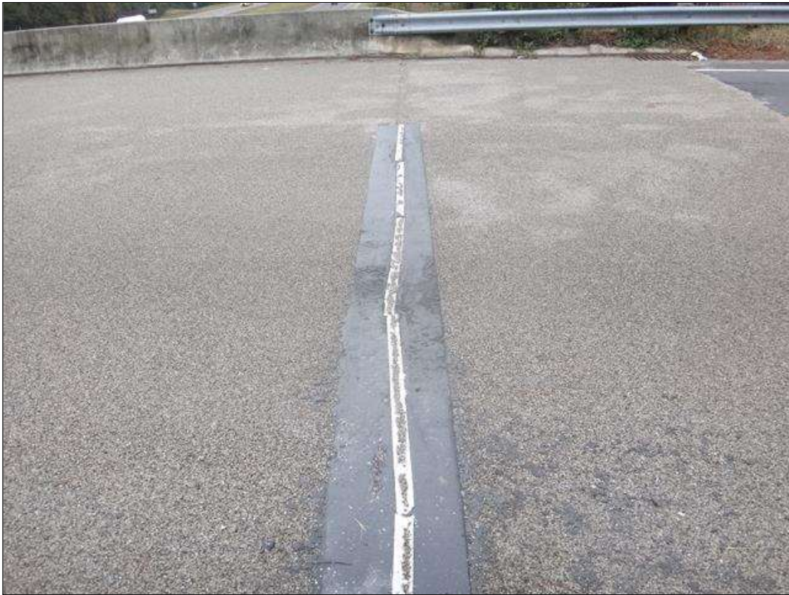
end bent 2 joint (partially covered with epoxy)
