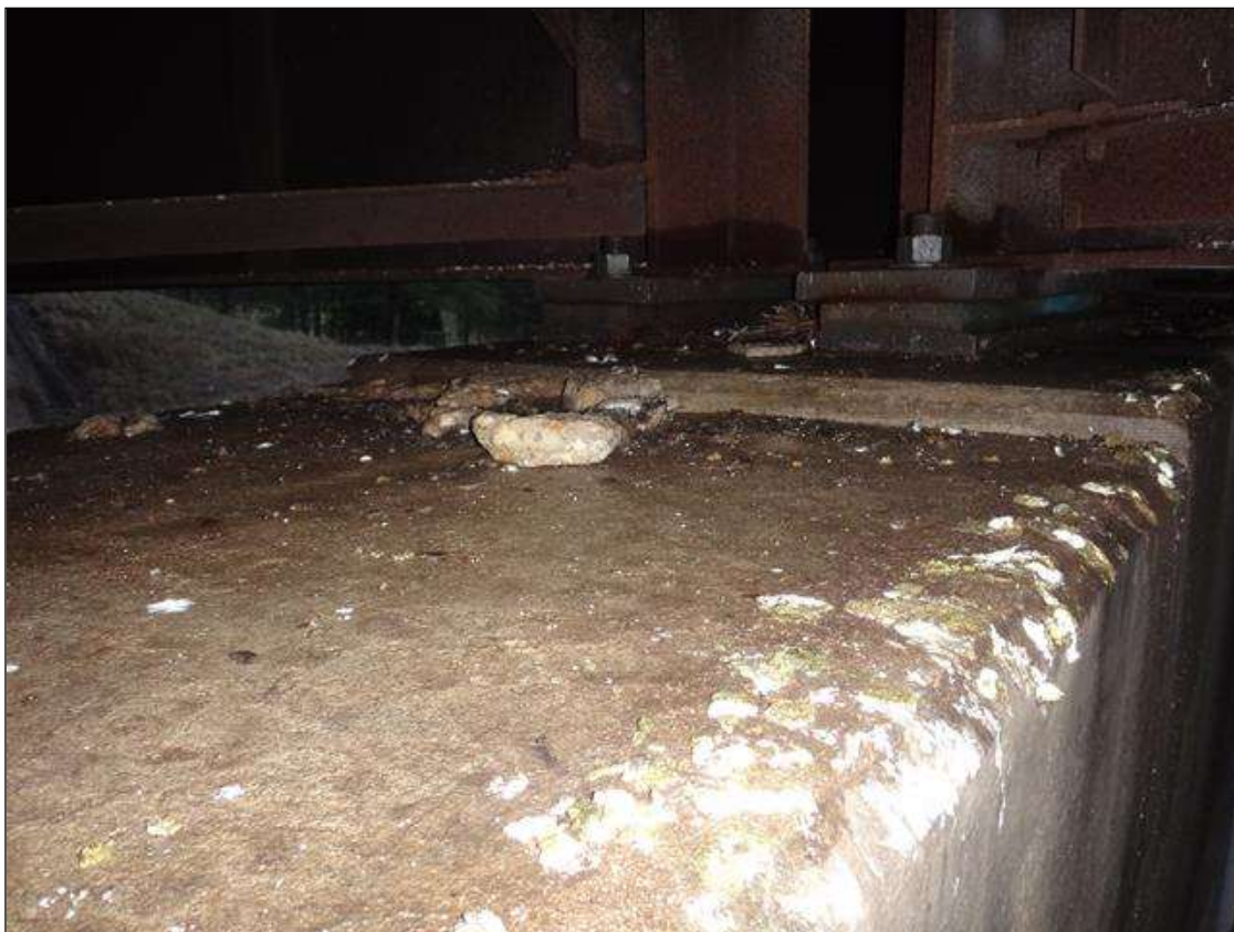
Bent 1 Cap: top of cap, debris accumulation (full length x full width)
