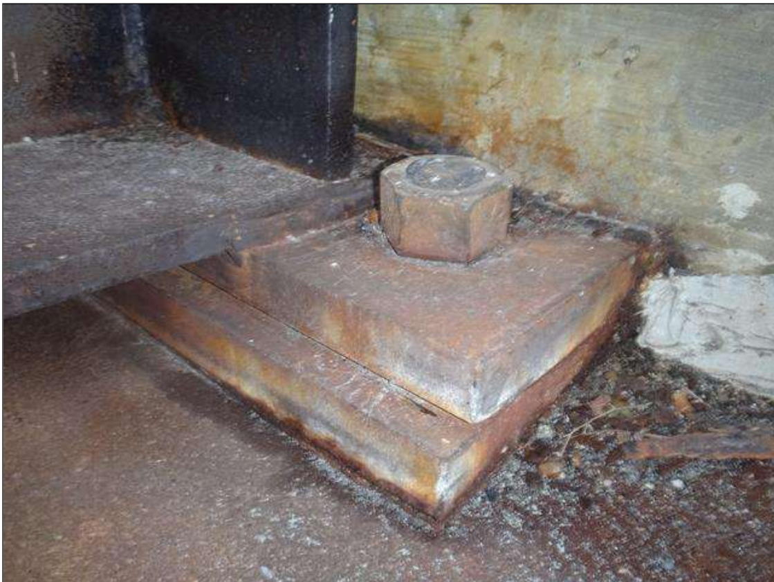
Span 2 Beam 6 Far Bearing: paint failure with surface rust
