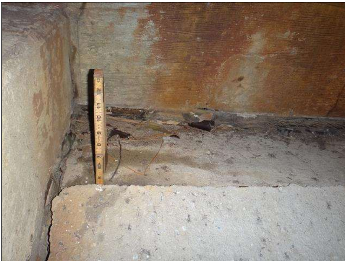
top face of slope protection below bay 5, seperated and settled (8ft x up to 3/4in x 5in) (photo 1 of 2)
