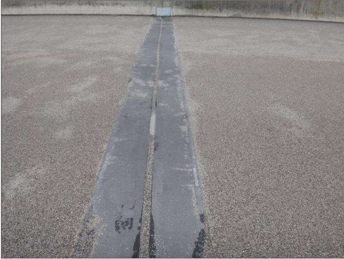
Expansion Joint 2: debris accumulation (full length)
