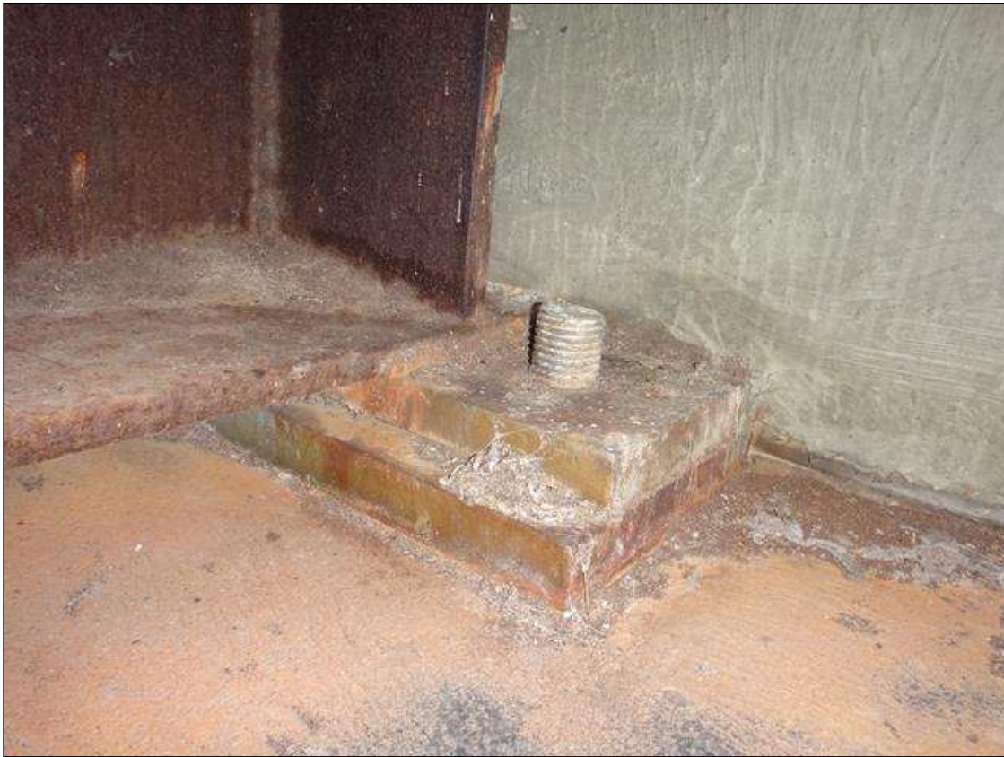
Span 2 Beam 2 Far Bearing: (2) anchor bolt nuts, missing
