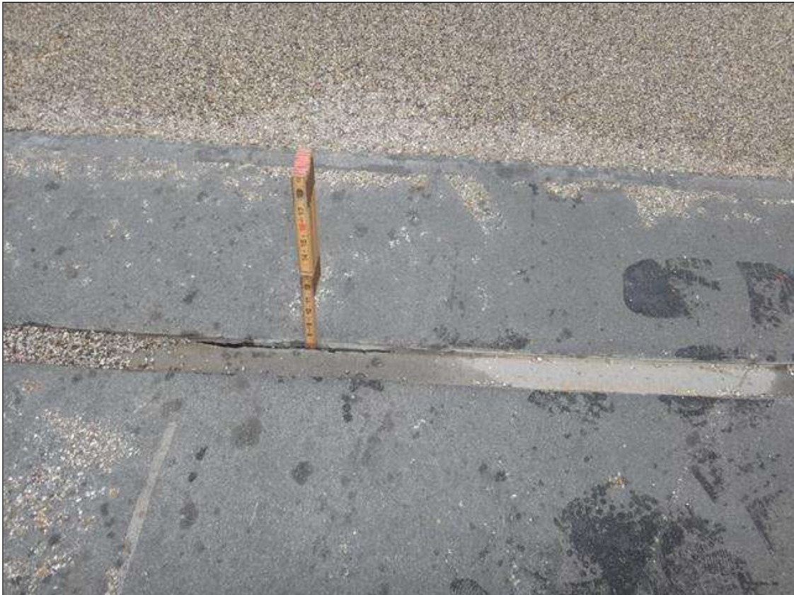
Expansion Joint 2: westbound lane at 10ft from rail, joint material separated from deck (1ft x 1/2in x full depth)
