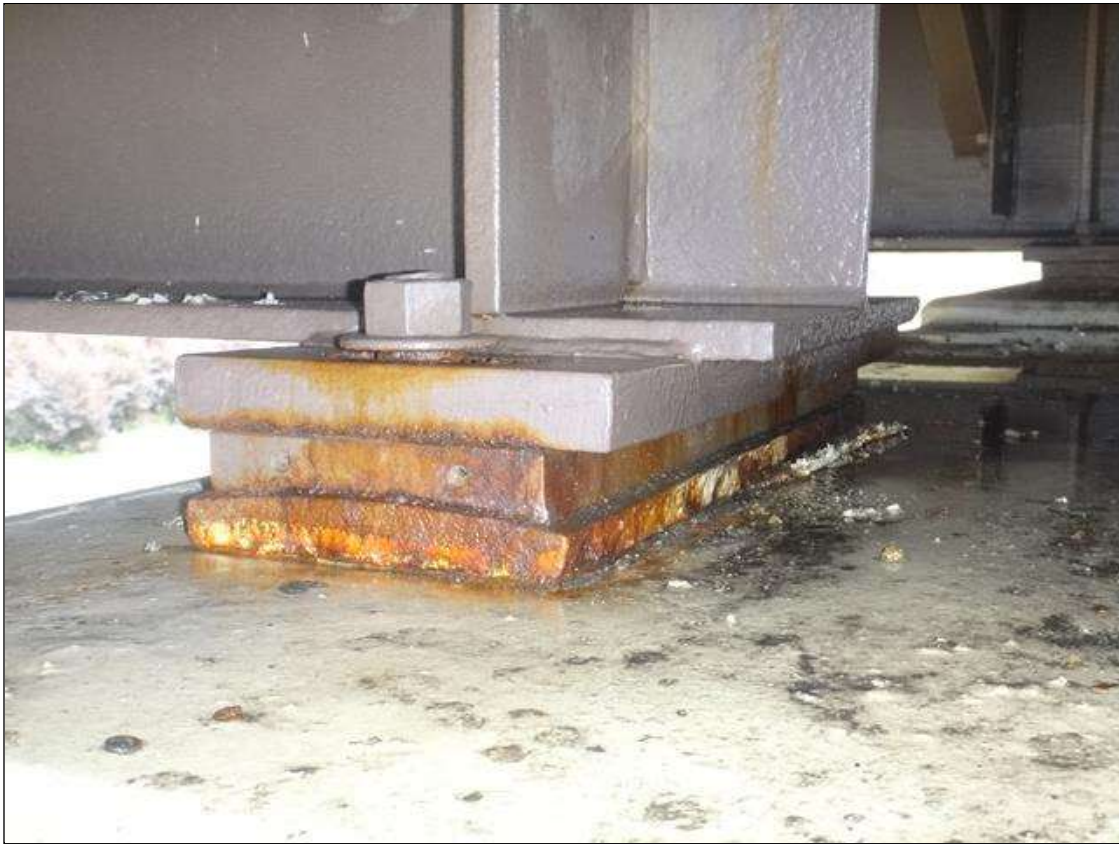
Span 2 Beam 2 Near Bearing: paint failure with surface rust
