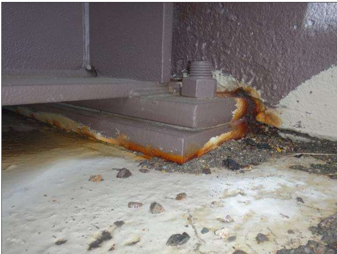
Span 2 Beam 9 Far Bearing: rust stains (3sf)
