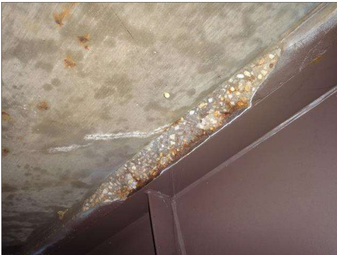
Span 2 Deck: underside bay 8 next to beam 9 at end bent 2, edge spall (30in x 4in x 1-1/2in) and adjacent diagonal crack (5-1/2ft x 1/32in) with efflorescence (photo 1 of 2)
