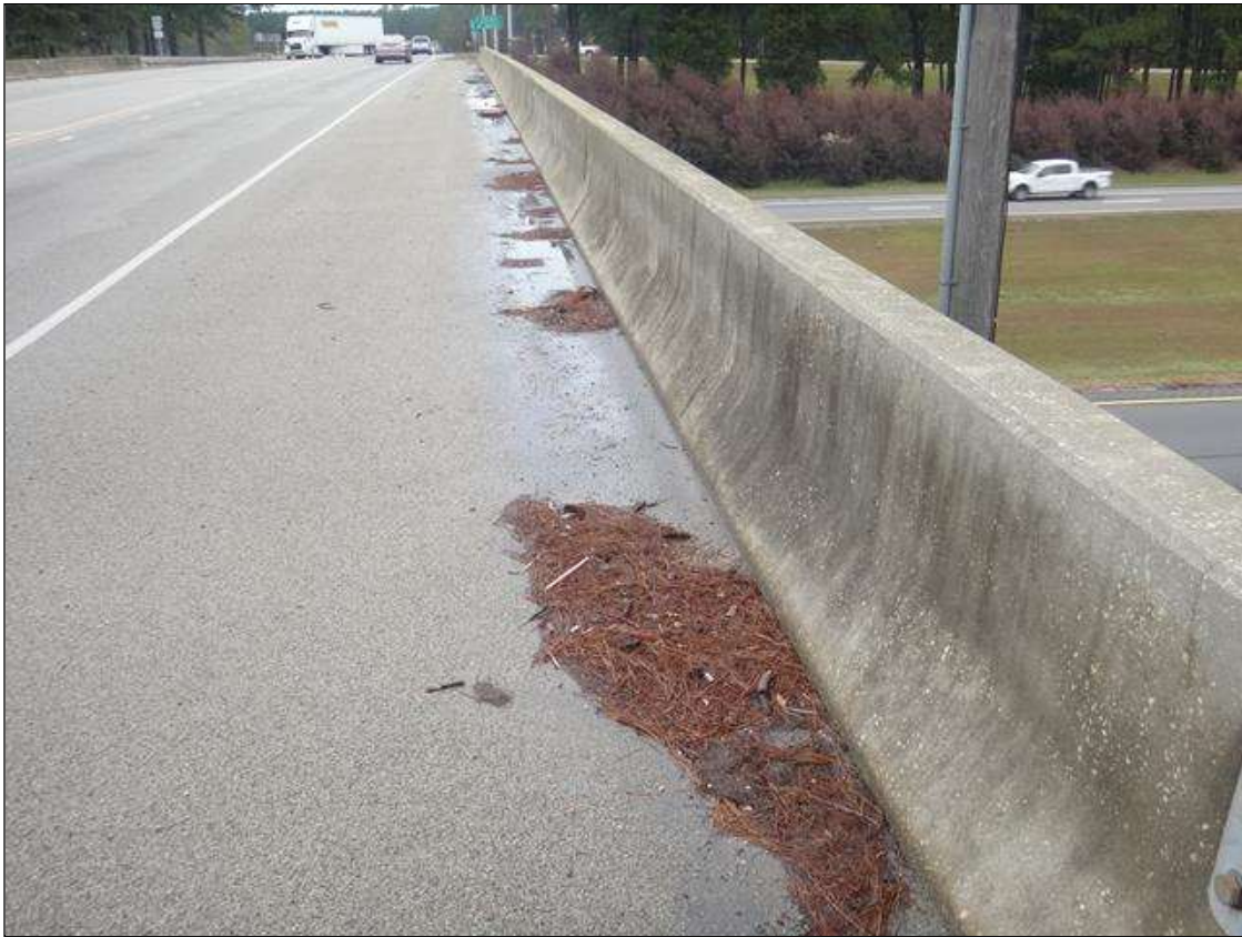
east shoulder, debris accumulation (full length x 3ft)
