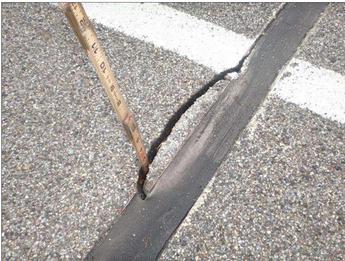
Expansion Joint 2 : west shoulder next to white line, broken section (1ft x 2in x up to 3in)
