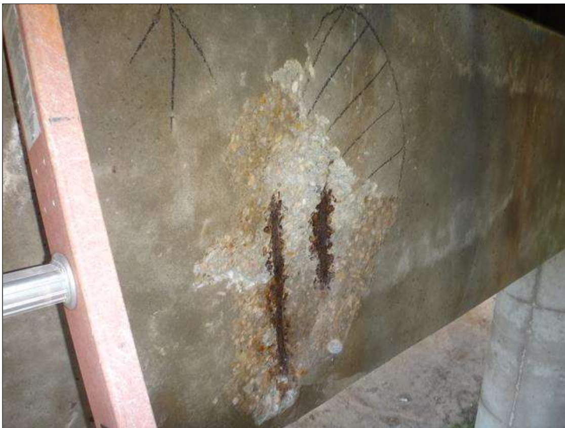
Bent 1 Cap 1: north face at bay 8, spall (2ft x 21in x up to 2in) with exposed rusted rebar and adjacent delamination (15in x 10in)
