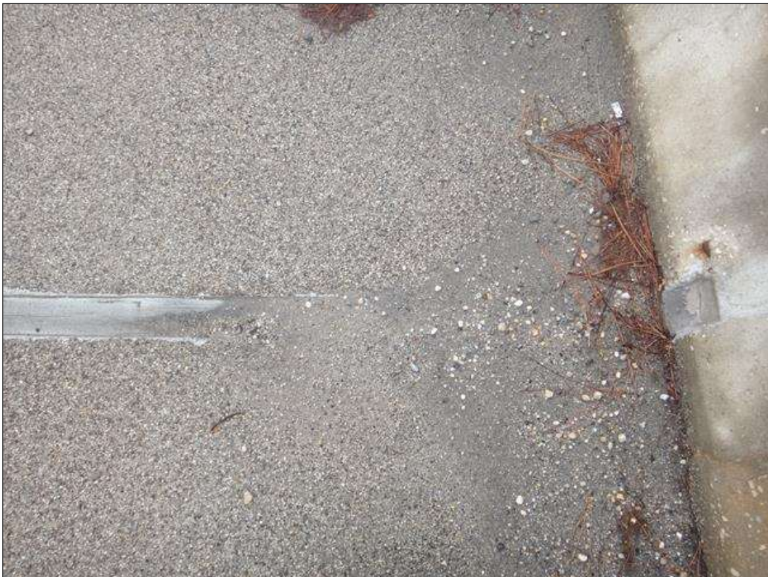
Expansion Joint 1 : east shoulder, debris accumulation (3ft)
