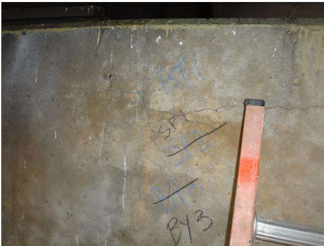
Bent 1 Cap 1: south face at bay 3, horizontal crack (30in x 1/16in) and vertical crack (15in x 1/16in)
