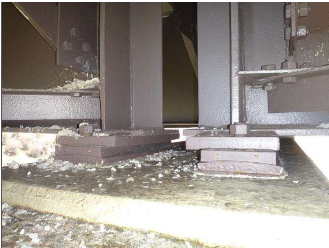
interior bearing assembly
