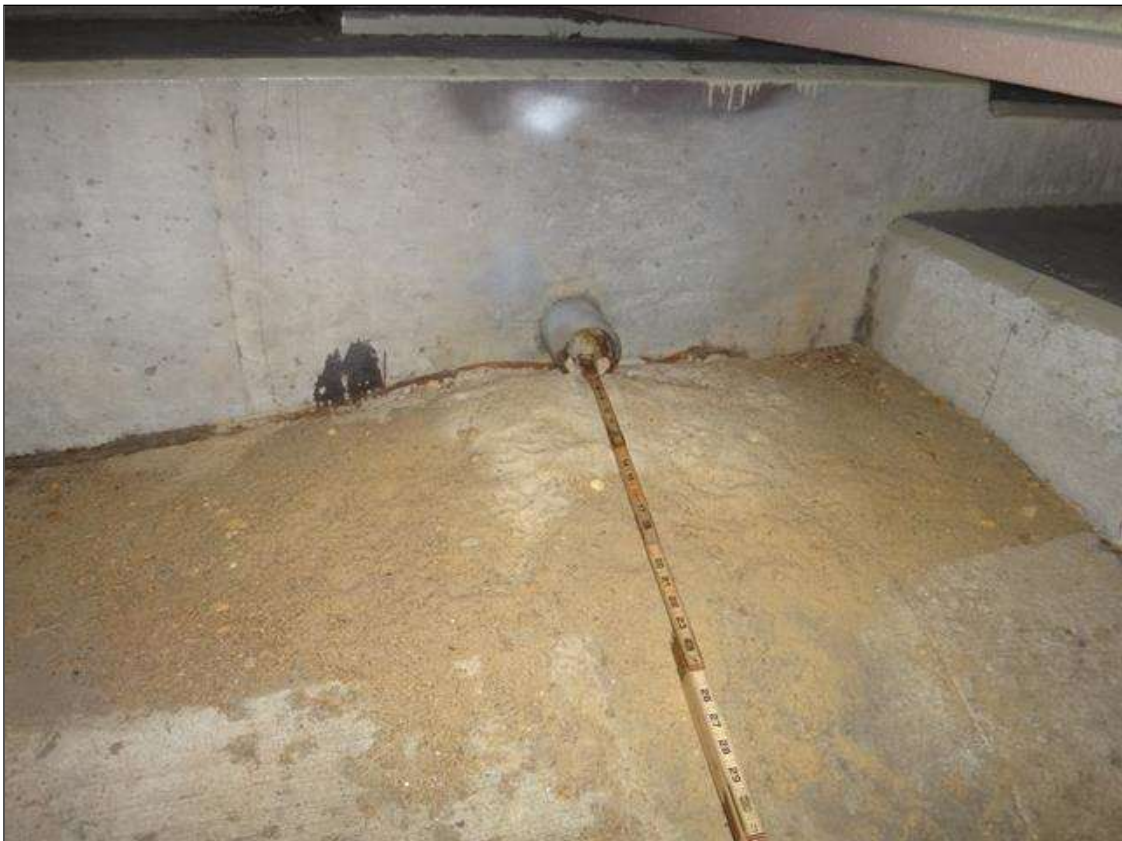
end bent 1 weepage holes under beams 4 and 5, partially blocked
