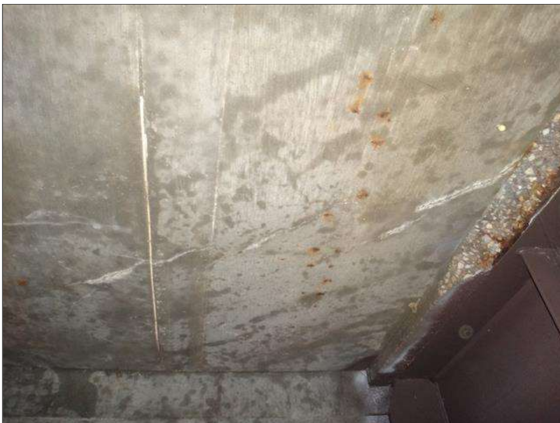
Span 2 Deck: underside bay 8 next to beam 9 at end bent 2, edge spall (30in x 4in x 1-1/2in) and adjacent diagonal crack (5-1/2ft x 1/32in) with efflorescence (photo 2 of 2)
