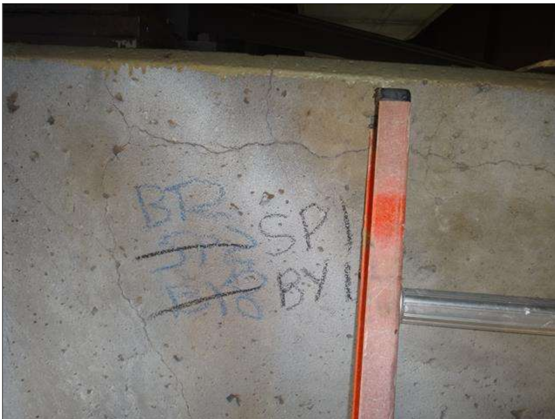
Bent 1 Cap 1: south face at bay 1, horizontal crack (2ft x 1/16in) and vertical crack (2ft x 1/16in)
