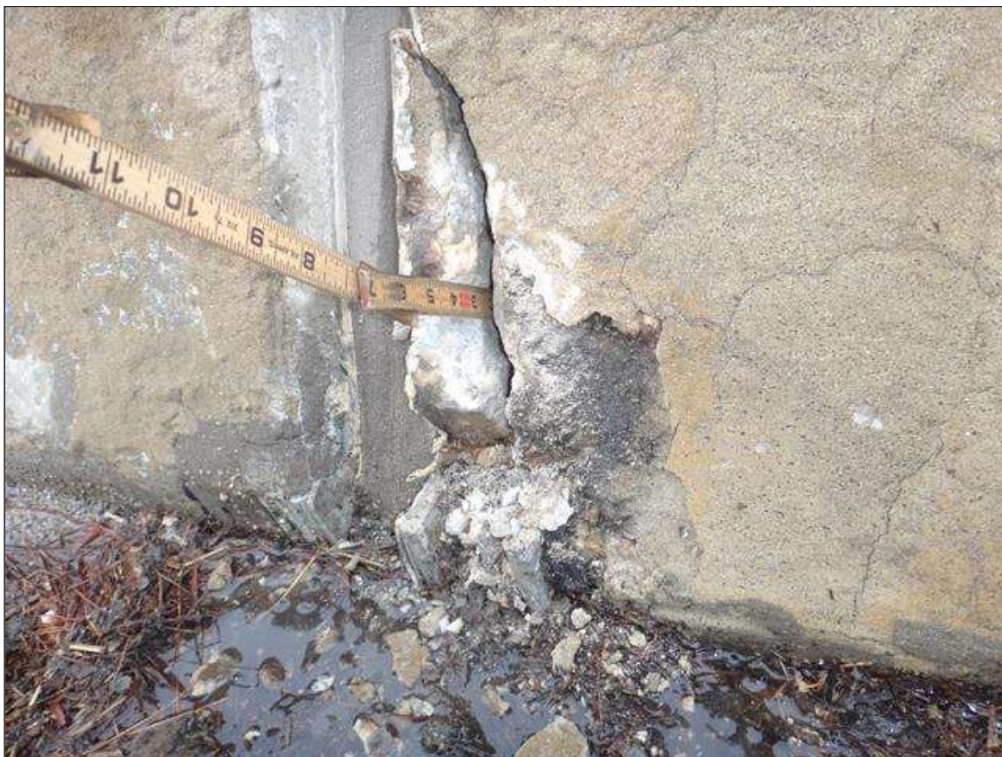
Span 1 Right Bridge Rail: base of rail at bent 1, spall (1ft x 6in x up to 3in)
