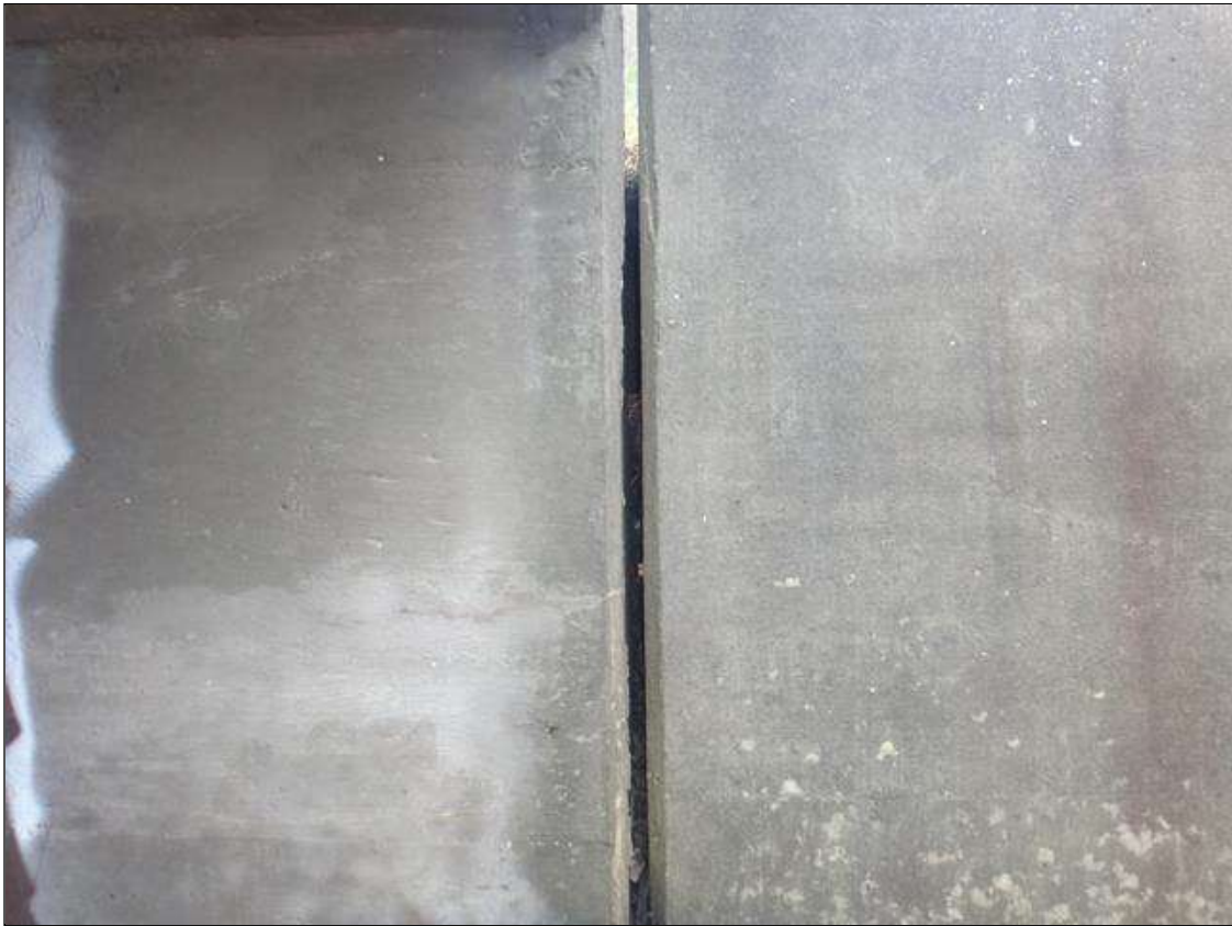
all wingwalls, missing joint material (full height)
