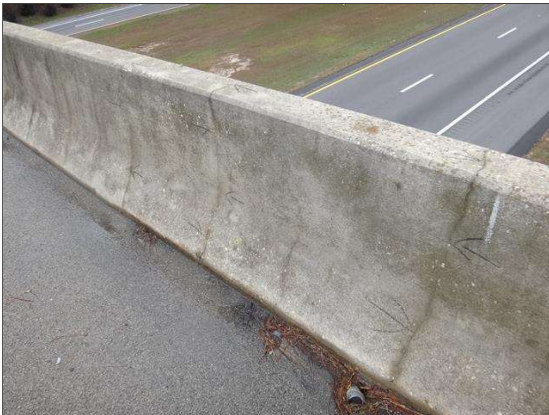
Span 2 Left Bridge Rail: scattered throughout at random, multiple vertical cracks (full height x hairline)
