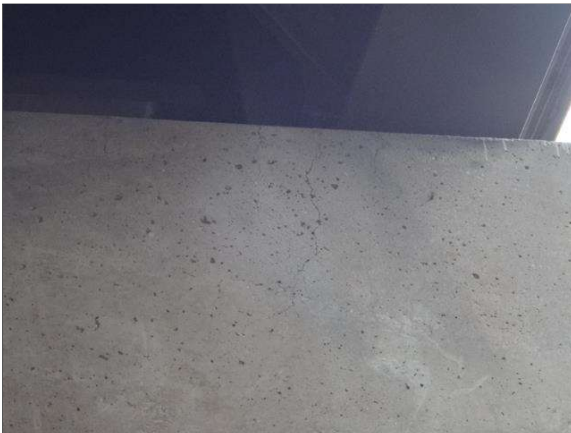
Bent 1 Cap 1: north face under beam 1, vertical crack (18in x 1/16in)
