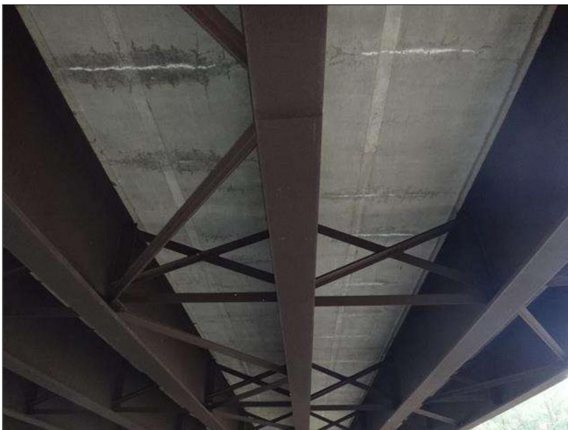
Span 2 Deck: underside scattered throughout at all bays, multiple transverse cracks (full width x hairline) with efflorescence
