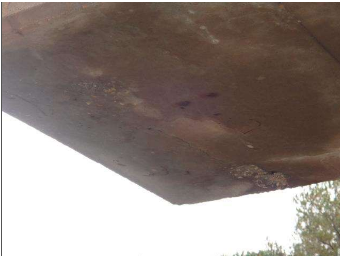
Bent 1 Cap 1: underside at east end, transverse crack (full width x 1/16in) and adjacent spall (6in x 3in x 1/4in)
