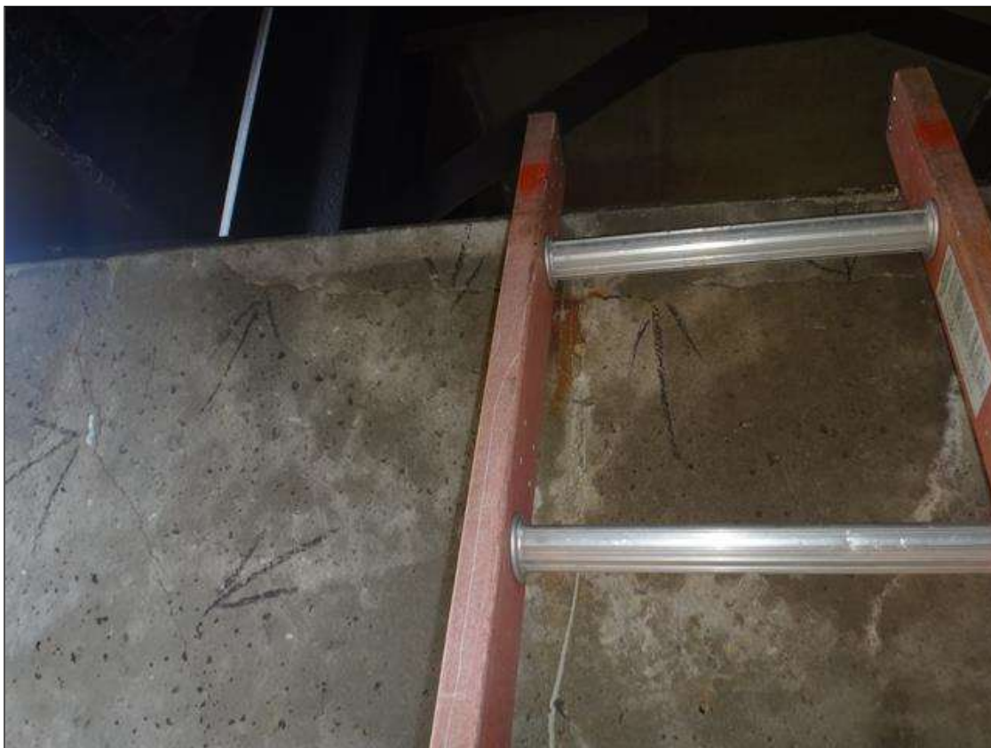
Bent 1 Cap 1: north face at bay 8, diagonal crack (18in x 1/16in) and horizontal crack (4ft x up to 1/8in)
