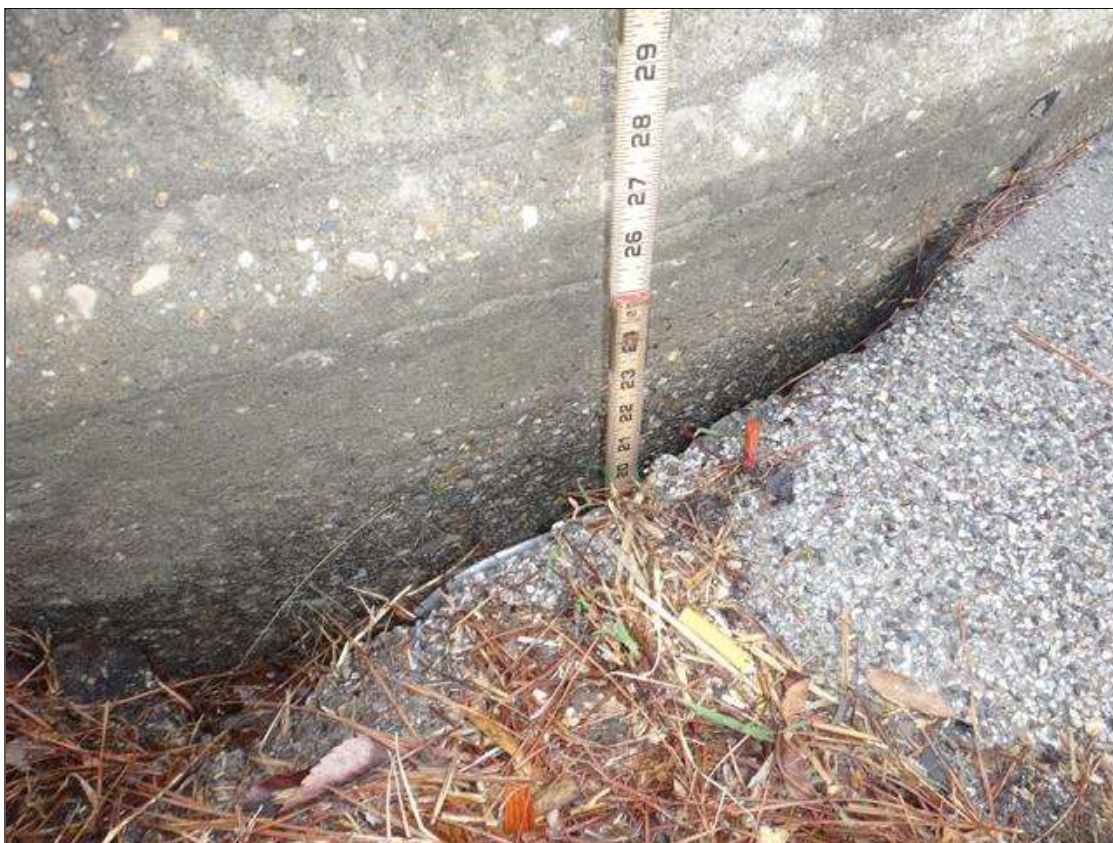
west shoulder between approach slab and left bridge rail at 2ft from end bent 1, erosion hole (2ft x up to 5in x up to 21in) (photo 2 of 2)
