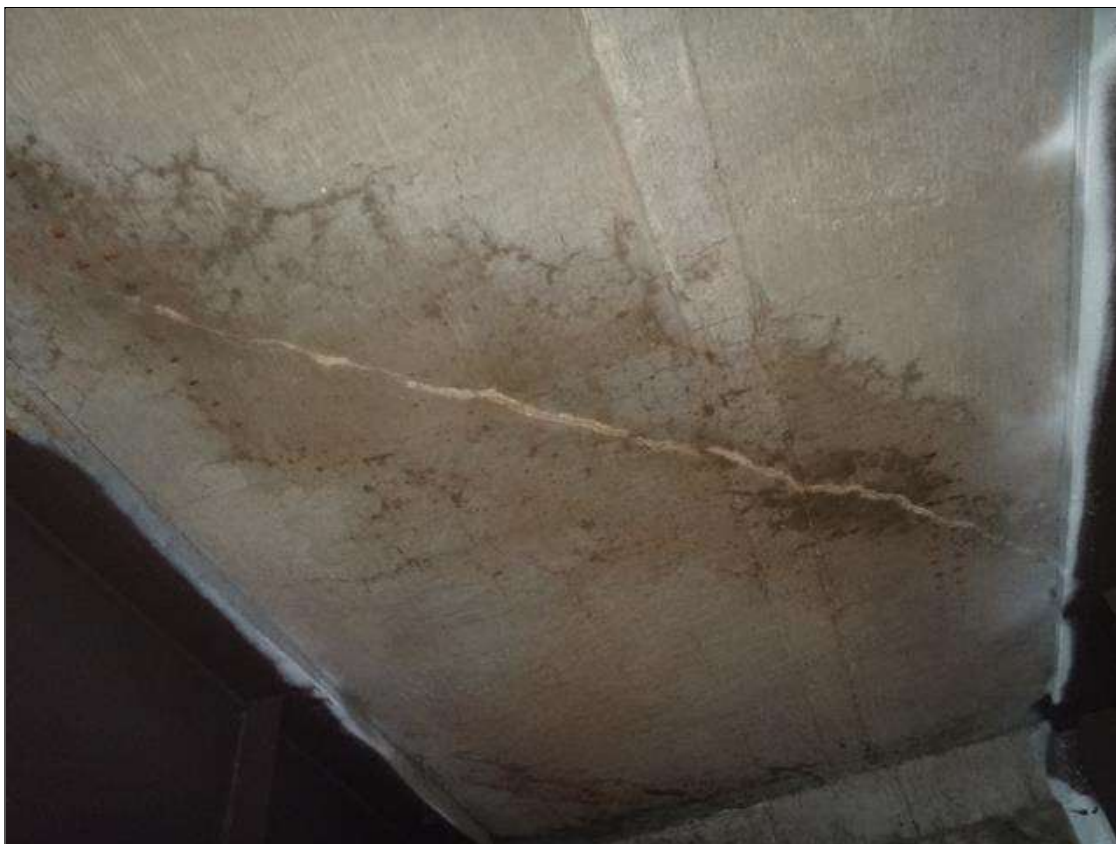
Span 2 Deck: underside bay 2 at end bent 2, diagonal crack (10ft x 1/32in) with efflorescence
