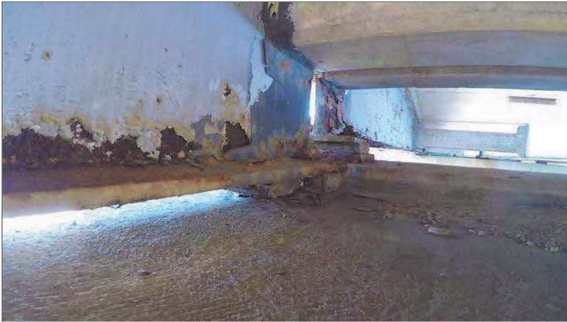
Span 4 Beam 4: Minor corrosion with pack rust initiating with minor section loss ( < 1/16 " ) on bottom 9" web and bottom flange for 1' at pier 3. Light surface rust on bottom of web and top and bottom flanges along full length of beam.
