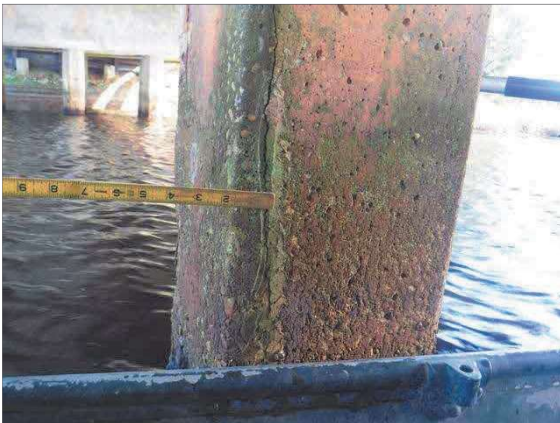
Bent 2 Pile 3: Up to 0.025" vertical cracks on west and north faces from waterline up 3'.
