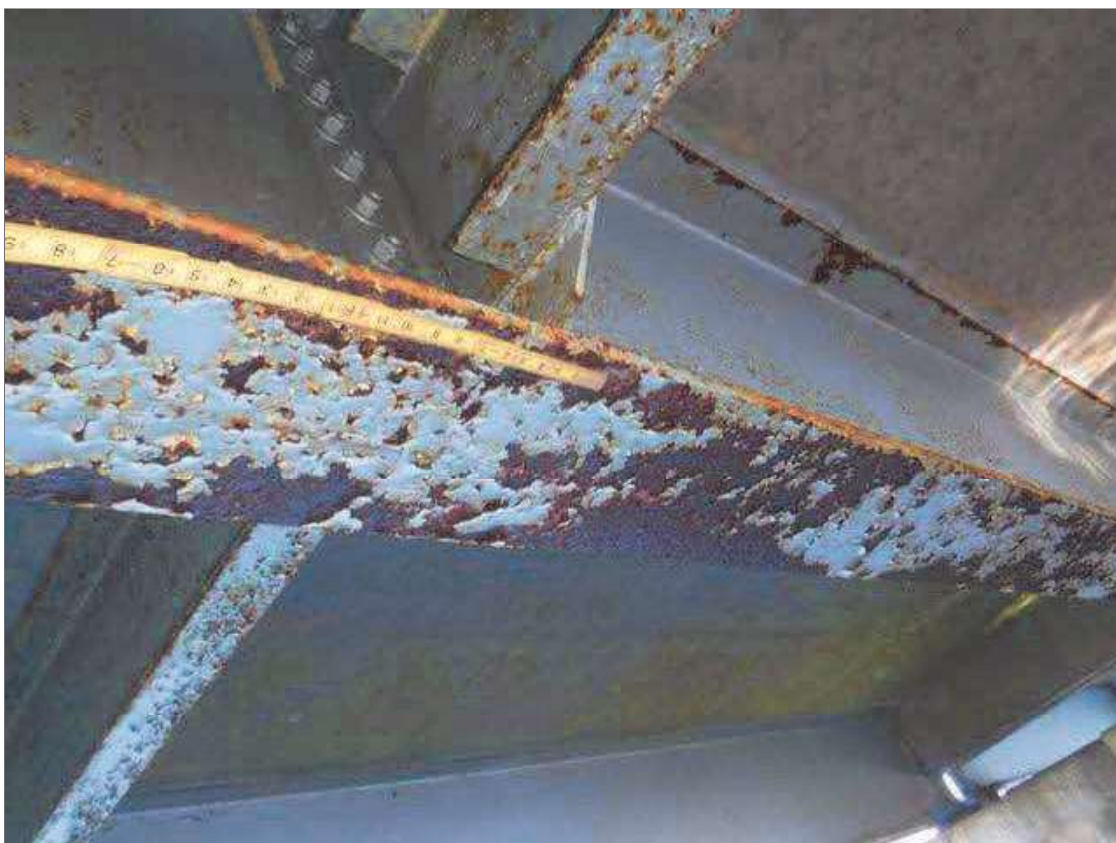
Span 1 Beam 2: Minor corrosion with pack rust initiating with no measurable section loss on bottom 9" web and bottom flange for 1' at pier 1. Light surface rust on bottom of web and top and bottom flanges along full length of beam.
