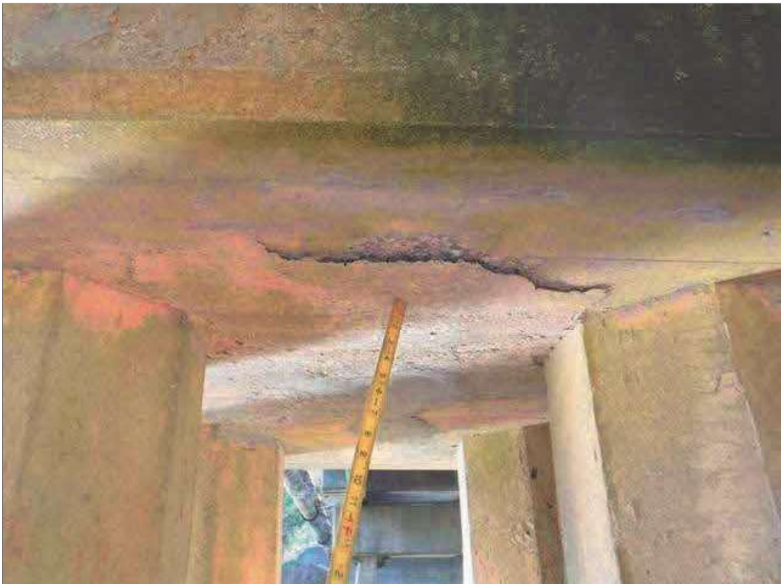
Bent 3 Cap 1: 18" X 21" AREA OF DELAMINATION IN BOTTOM OF CAP BETWEEN PILES 6 AND 8
