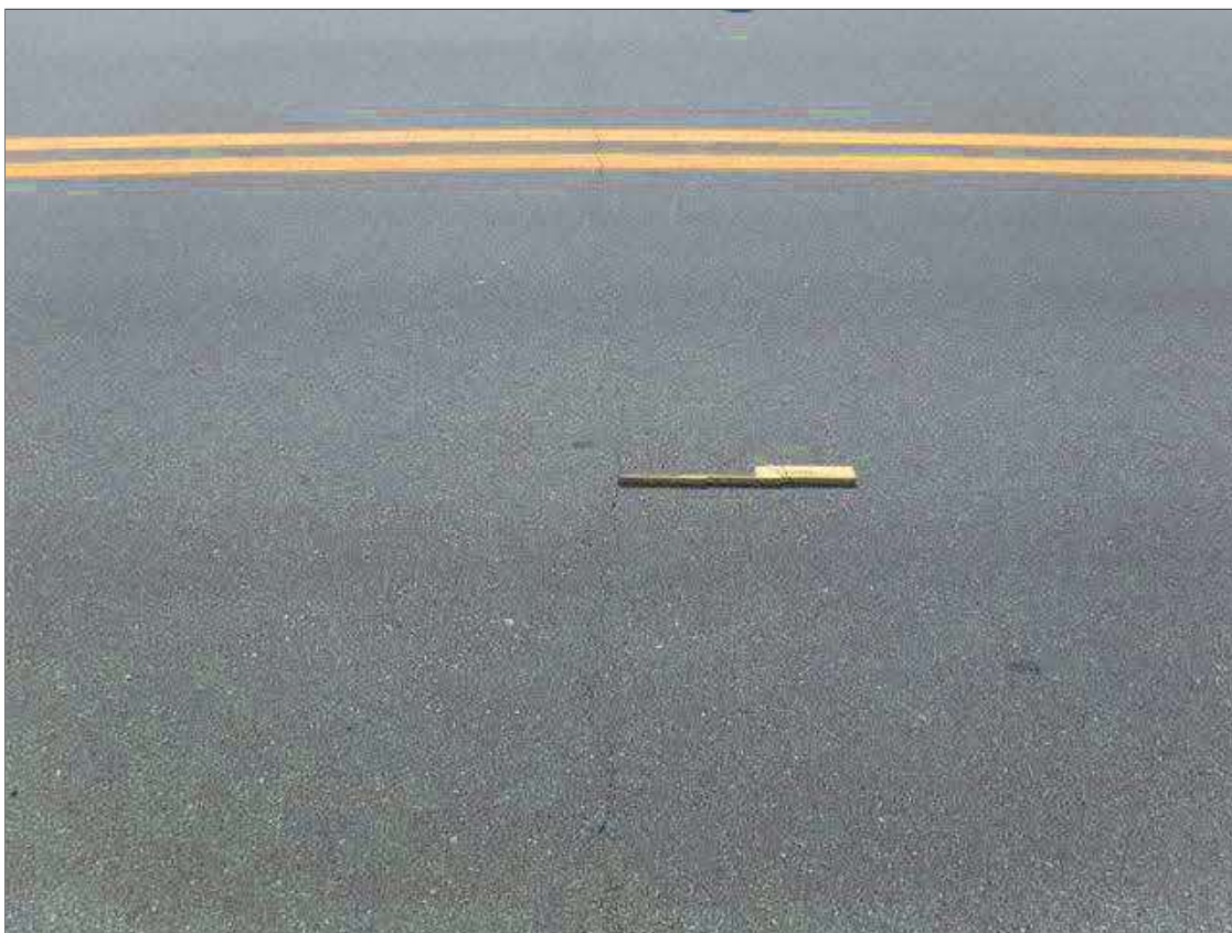
Span 3 Wearing Surface: UP TO 1/16" TRANSVERSE CRACK ALONG BENT 2
