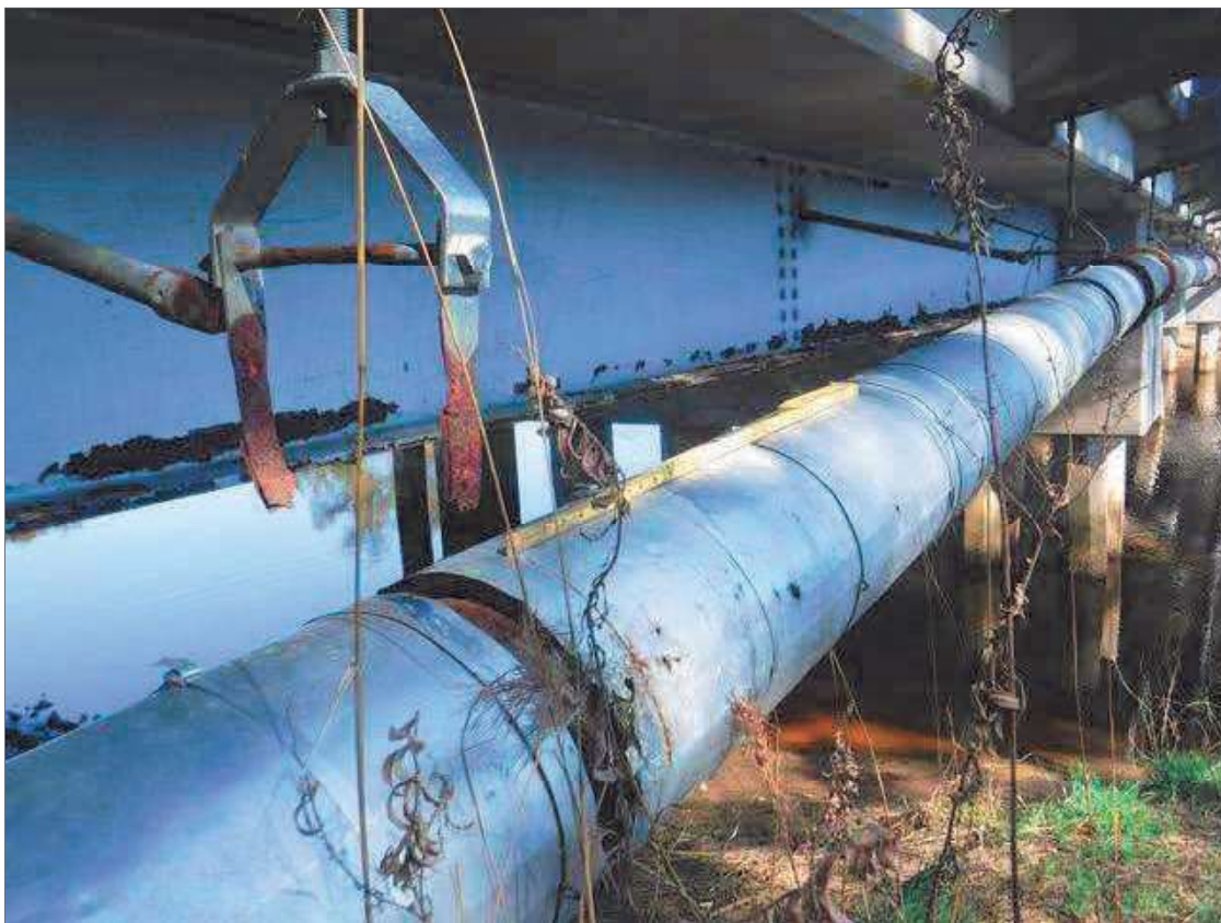
(2) BROKEN UTILITY HANGERS ATTACHED TO RIGHT OVERHANG AND BEAM 4 NEAR END BENT 1
