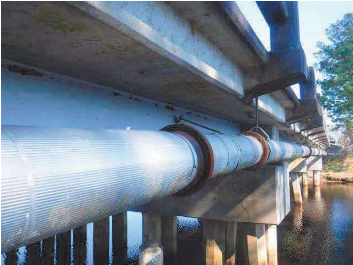
12" DIAMETER INSULATED DUCTILE IRON PIPE ATTACHED TO BOTTOM OF RIGHT OVERHANG AND BEAM 4
