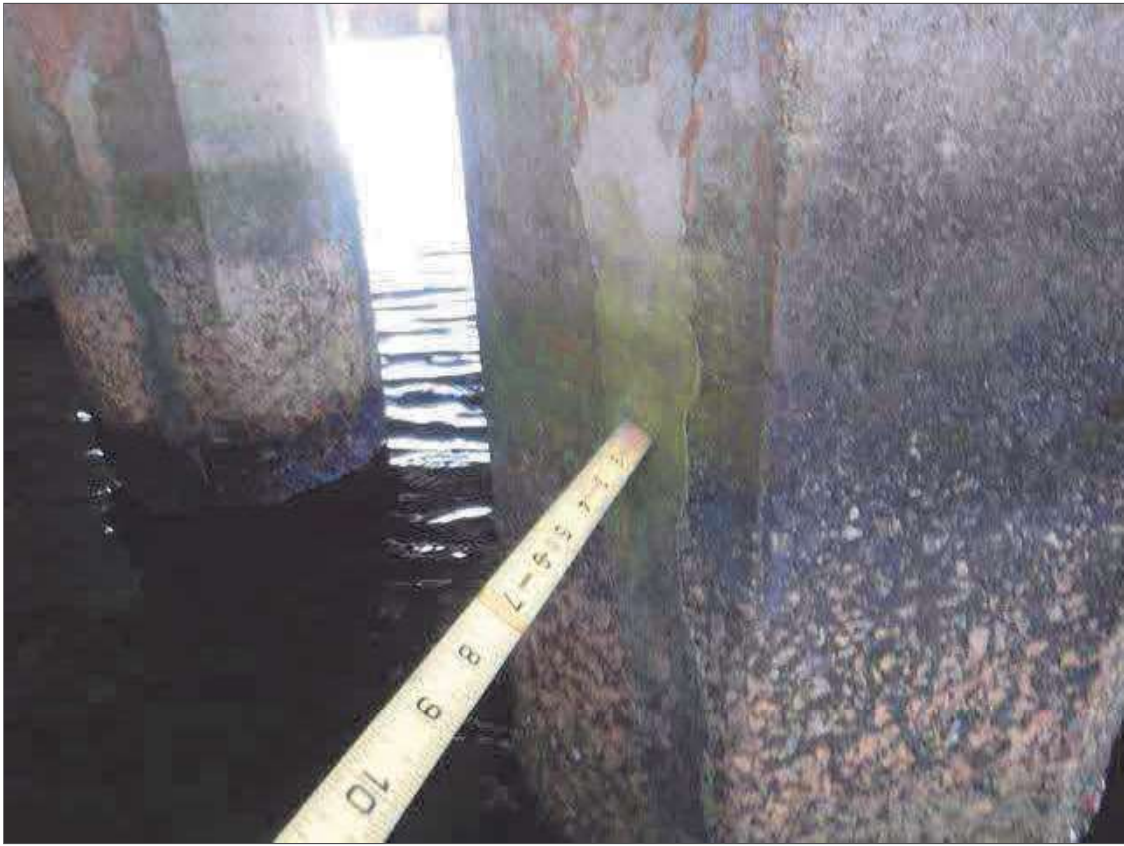
Bent 3 Pile 1: Vertical cracks on faces 5, 6 & 7 have been sealed.
