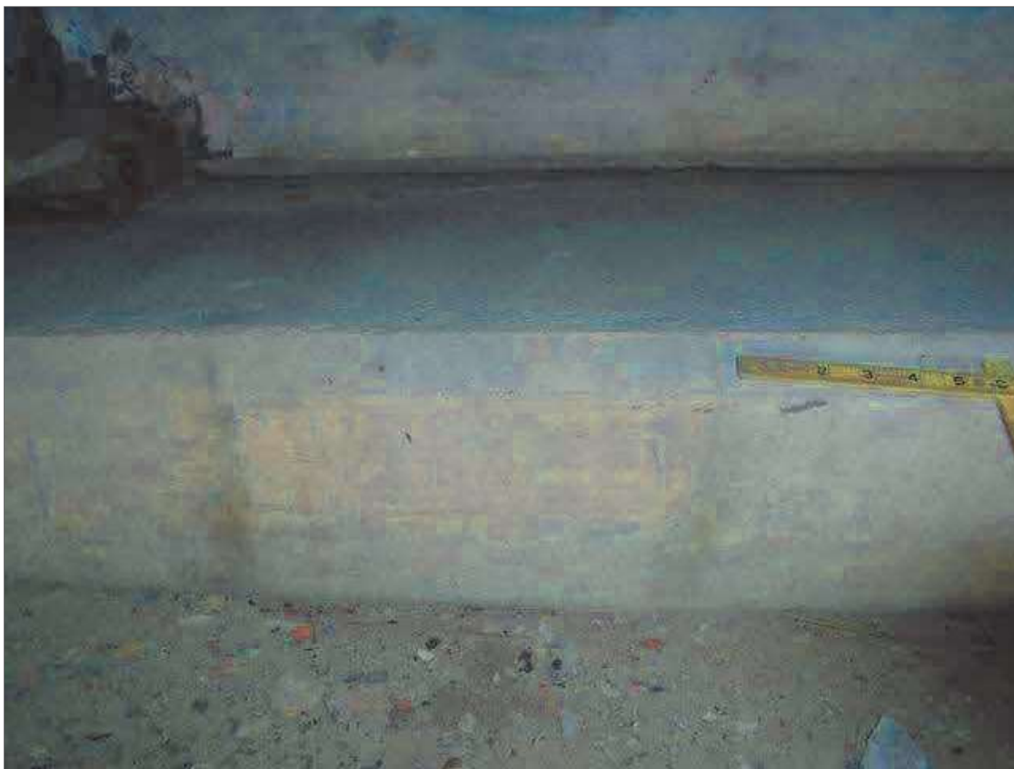
End Bent 1 Cap 1: Several hairline cracks at various locations along the top and front face of cap.
