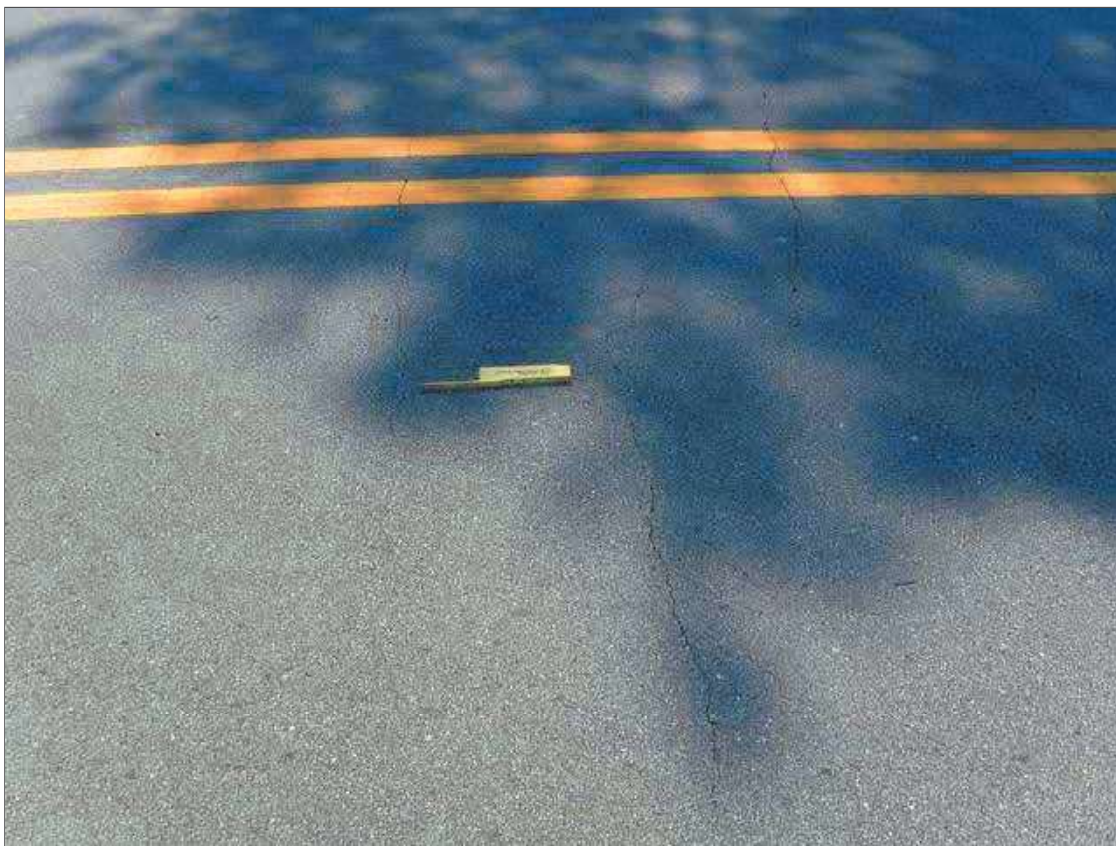
Span 1 Wearing Surface: UP TO 1/16" TRANSVERSE CRACK ALONG END BENT 1 FILL FACE IN WESTBOUND LANE
