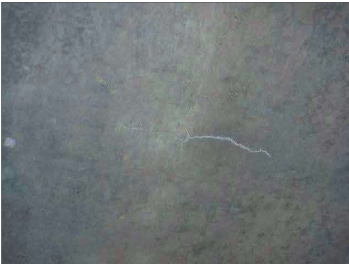
Span 1 Deck: UP TO 0.012" TRANSVERSE CRACKS WITH EFFLORESCENCE IN VARIOUS LOCATIONS THROUGHOUT BOTTOM OF DECK
