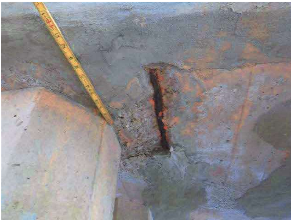
Bent 1 Cap 1: (2) FAILED PATCHES WITH UP TO 36" X 12" AREA OF DELAMINATION AND UP TO 14" X 7" X 1" DEEP SPALL WITH EXPOSED REBAR IN BOTTOM OF CAP AT PILE 5
