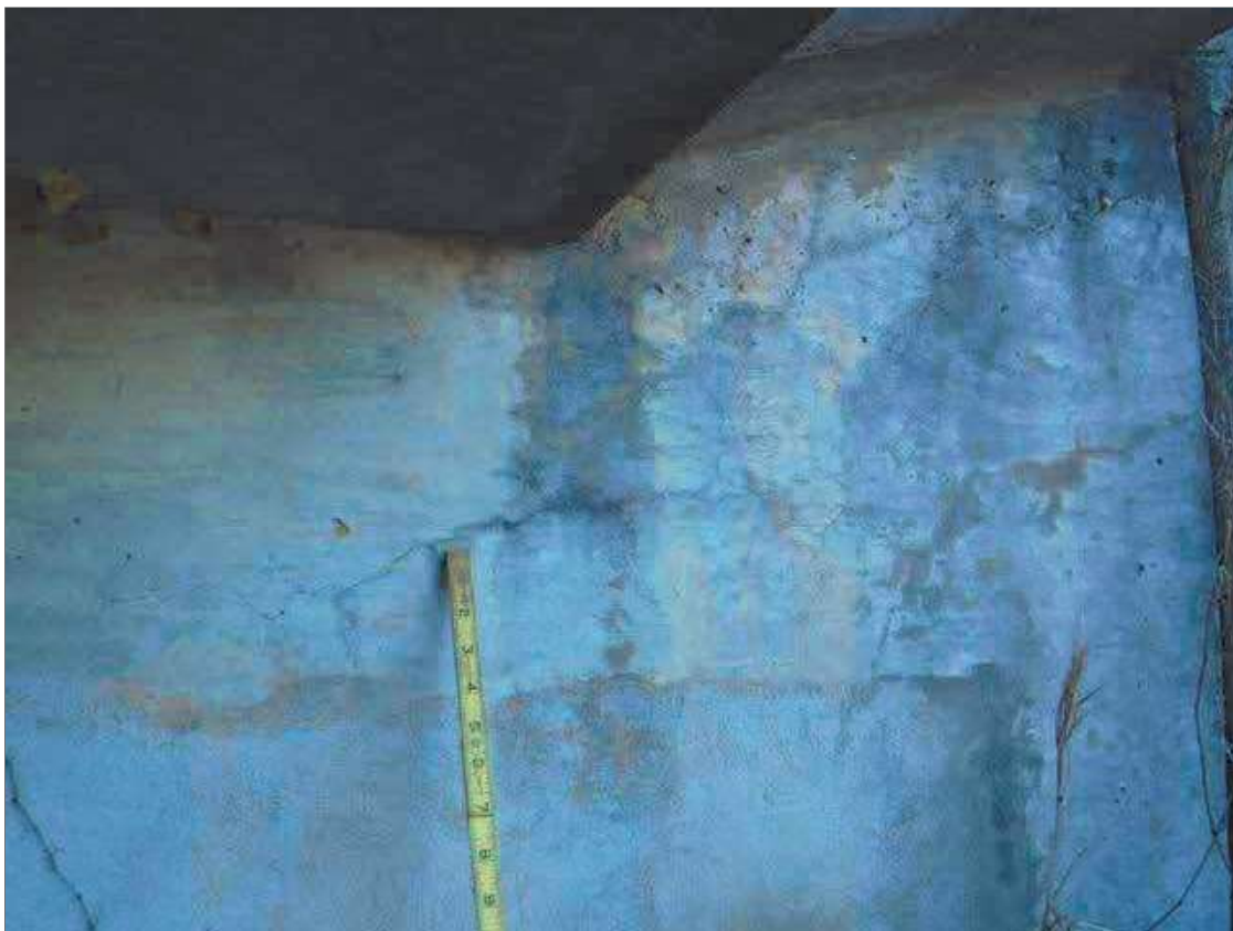
End Bent 1 Abutment: Hairline map cracking in on north end near wing wall
