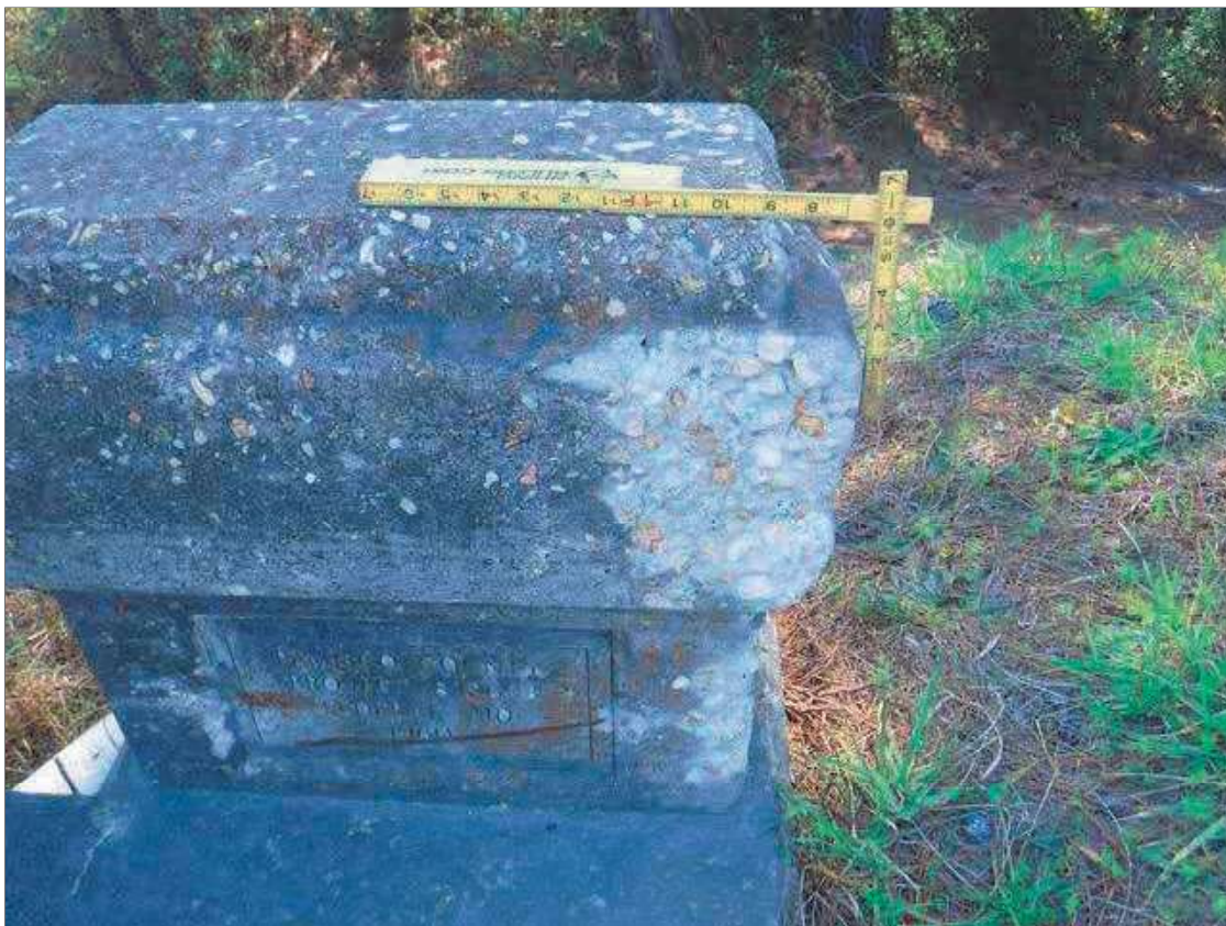
Span 1 Right Bridge Rail: 18" X 8" X 1" DEEP SPALL IN FACE OF END POST AT END BENT 1
