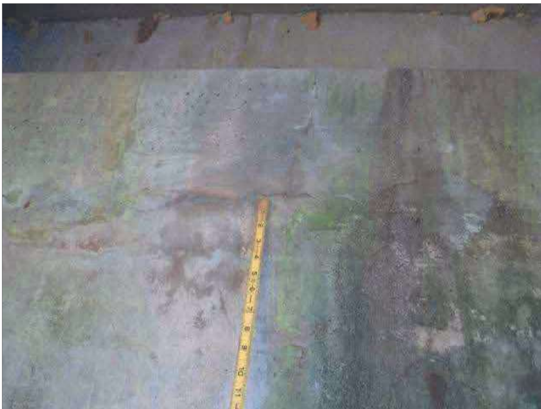
Bent 3 Cap 1: 30' OF UP TO 0.012" HORIZONTAL CRACKS IN SPAN 2 FACE OF CAP
