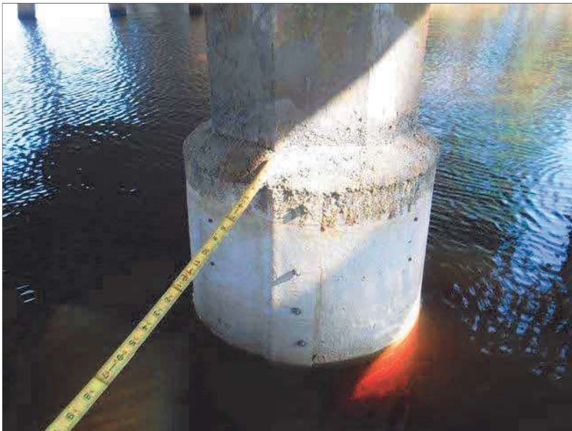
Bent 1 Pile 5: Hairline to 1/64" vertical cracks on faces 1, 2 & 8 from waterline up 4'.
