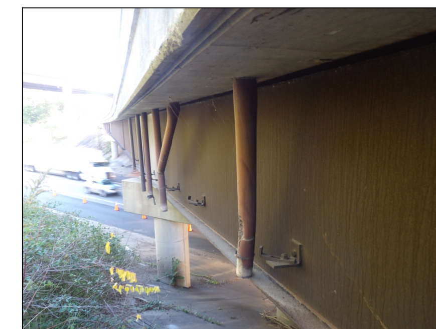
SPAN C - 2 DAMAGED DRAIN PIPES
