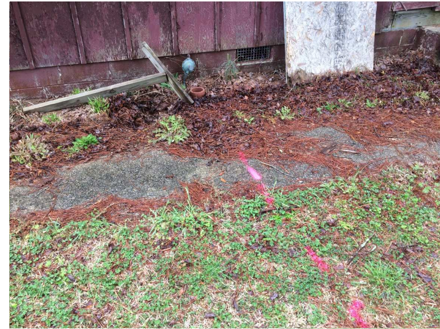
B. Approximate location of line leading from shop building to propane UST on south side of building.
