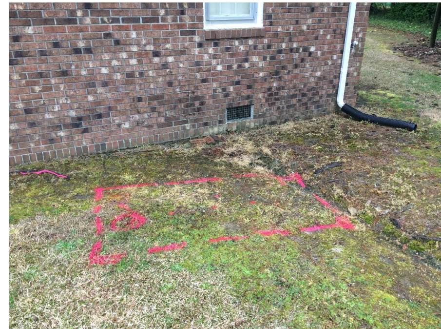
B. One probable UST marked near southwest corner of house. The probable UST is approximately 3 ft diameter x 6 ft long. The circle on the left side of the photo marks an apparent open fill port.
