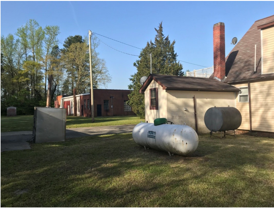
Photograph 5: View of the ASTs in the rear of the residence.
