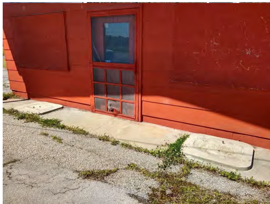
C. Close-up view of old dispenser pedestal locations on the front of the building.
