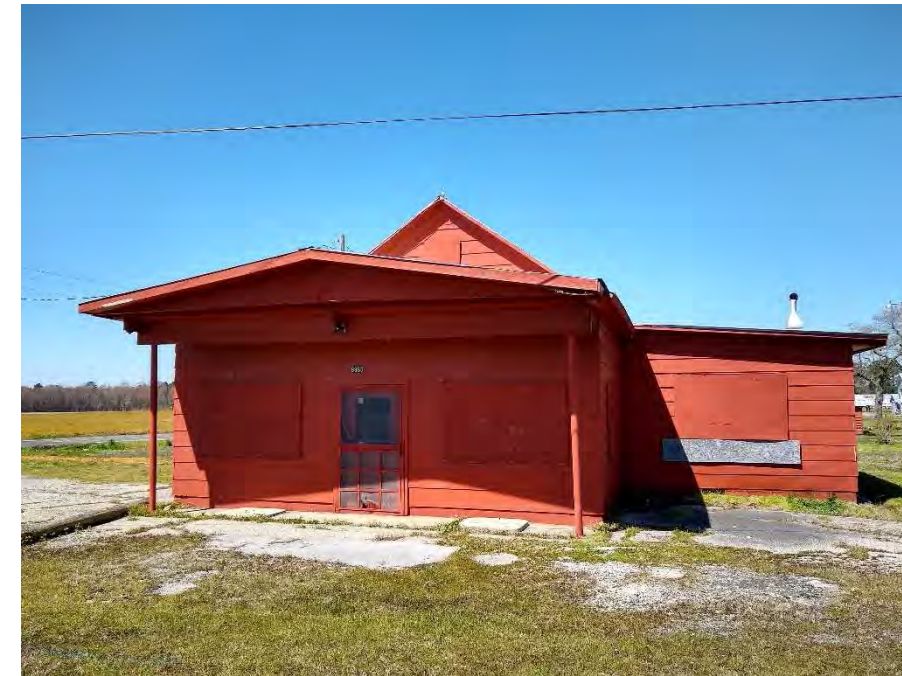
B. Front of former gas station building, photograph taken looking west. Note relic concrete pads on porch from former dispenser locations.
