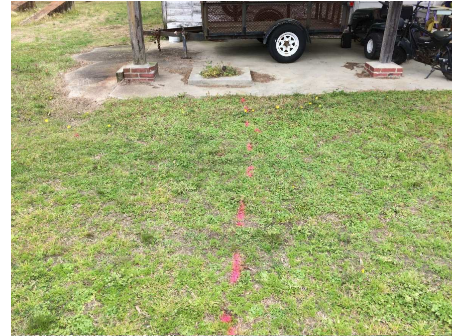
B. Possible relic product line leading west from pipe in middle of former dispenser pedestal, looking west.
