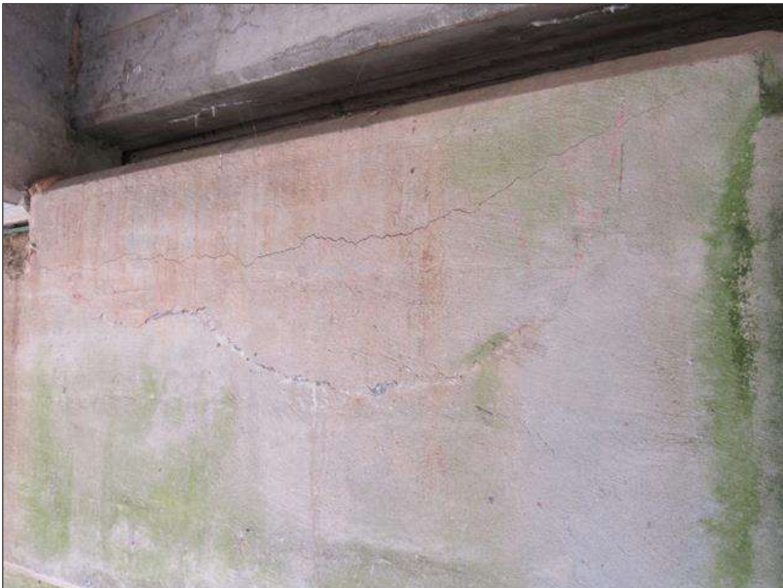
BENT 3 CAP, FAR FACE - DELAM (5SF) ABOVE COLUMN 1
