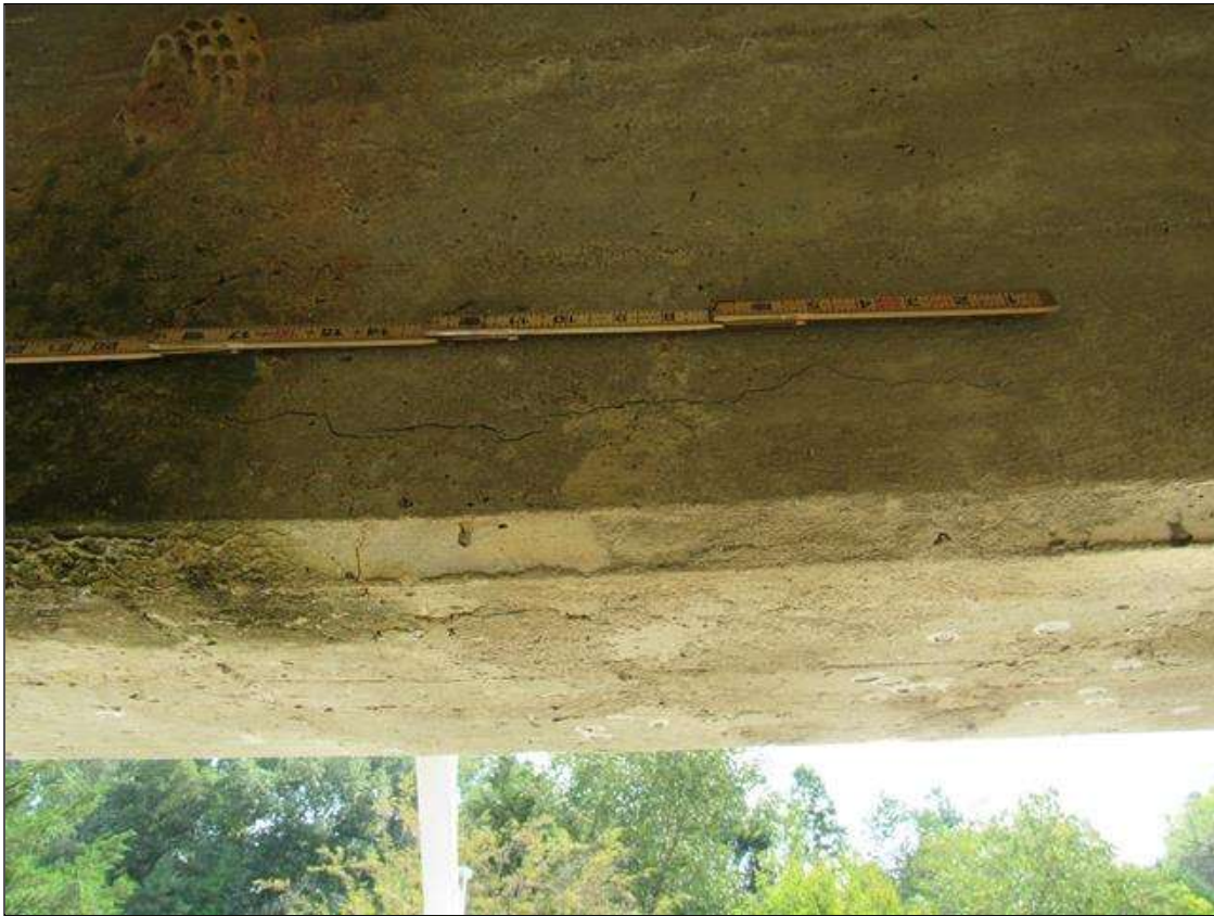
SPAN 4, BEAM 5 - DELAM (20IN X 5IN) BOTTOM LEFT EDGE NEAR MID-SPAN
