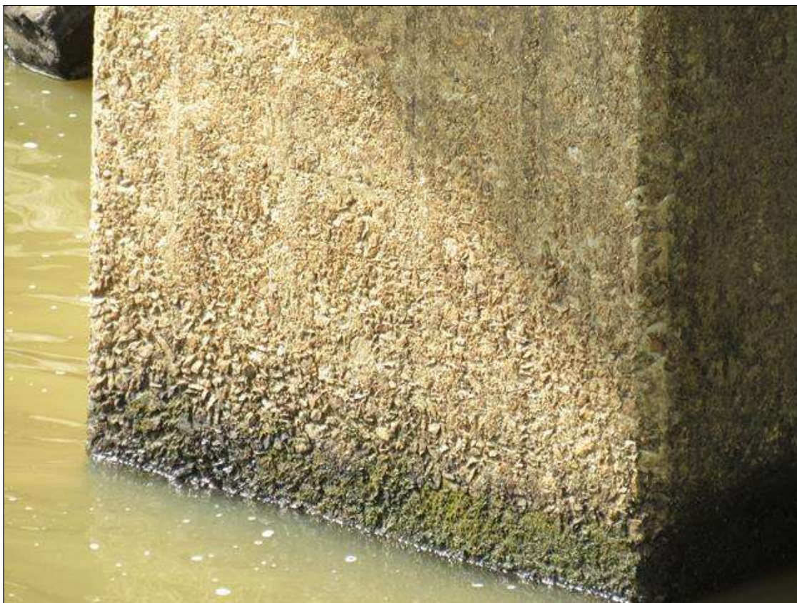
TYPICAL WATER SCALING, (UP TO 2FT H.) THROUGHOUT COLUMNS AT WATERLINE, BENT 1 COLUMN 1 FAR FACE
