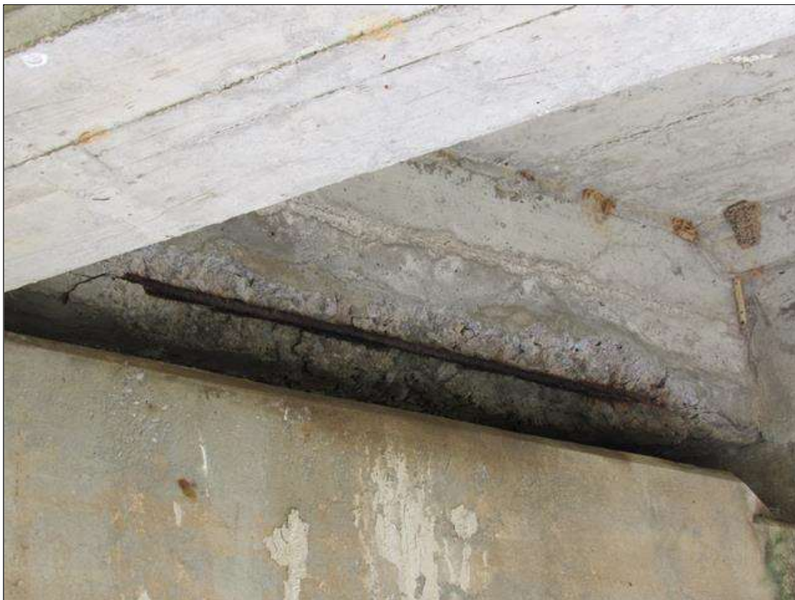
SPAN 2 FAR END DIAPHRAGM, BAY 4 - SPALL (4FT X 6IN X 3IN) WITH EXPOSED REINFORCING
