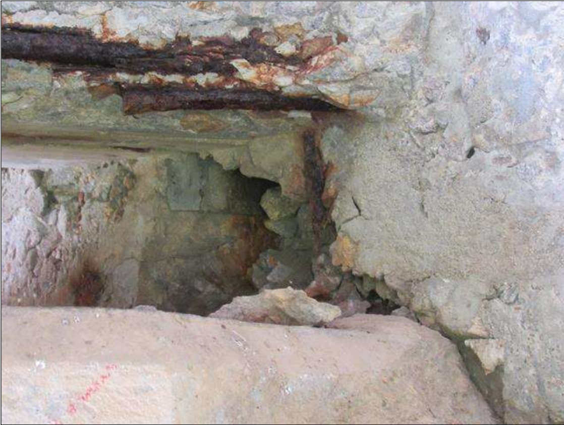
SPAN 5 BEAM 3 - SPALL (8IN X 6IN X 5IN) WITH EXPOSED REINFORCING, RIGHT SIDE NEAR END
