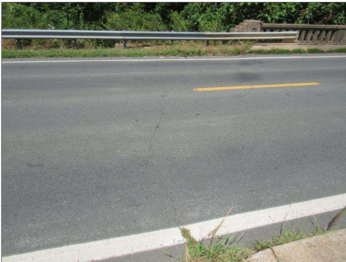
NEAR APPROACH & AWS OVER END BENT 1 - INTERMITTENT TRANSVERSE OPEN CRACKING, (UP TO 1/4IN X FULL L.) THROUGHOUT, FAR APPROACH SIMILAR
