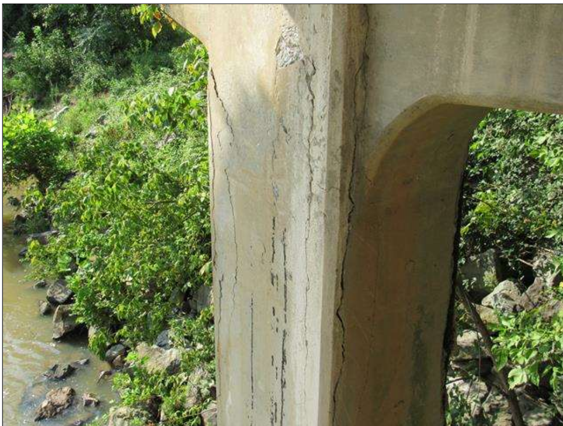
BENT 1 COLUMN 2, FAR FACE - (X2) DELAM (UP TO 7FT X 1FT) FAR LEFT & RIGHT CORNERS, STARTING AT BOTTOM OF CAP
