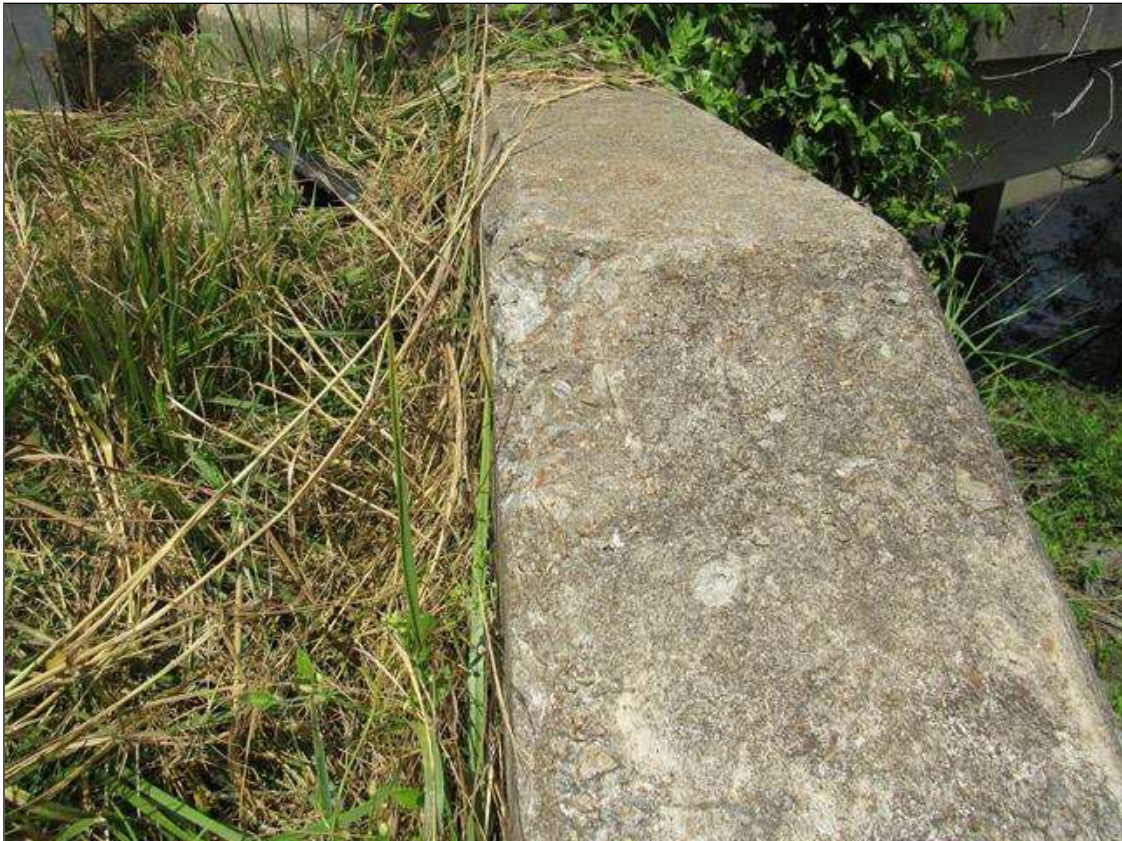
NEAR RIGHT WINGWALL - SPALL (10IN X 6IN X 1IN) NO EXPOSED REINFORCING, NEAR CORNER
