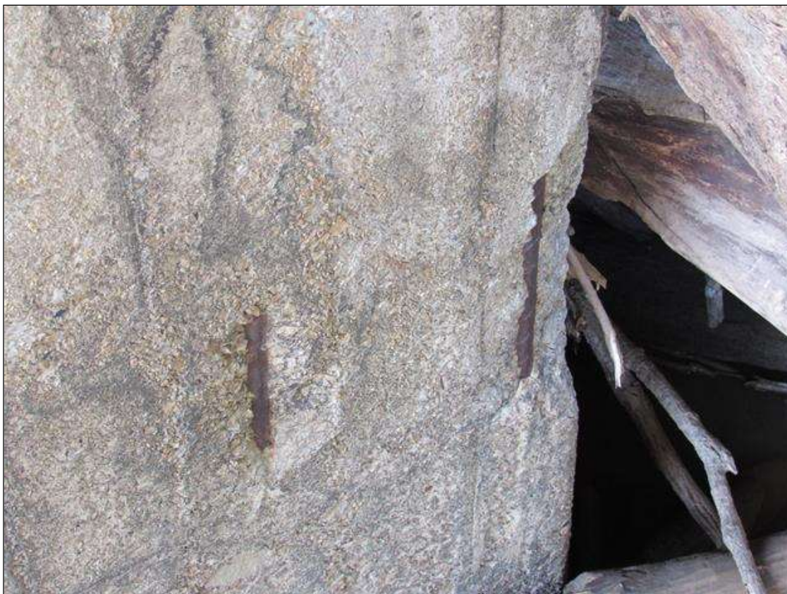
BENT 4 COLUMN 1 - (X2) SPALLS (UP TO 3FT X 8IN X 3IN) WITH EXPOSED REINFORCING, FAR LEFT CORNER 4FT FROM WATERLINE
