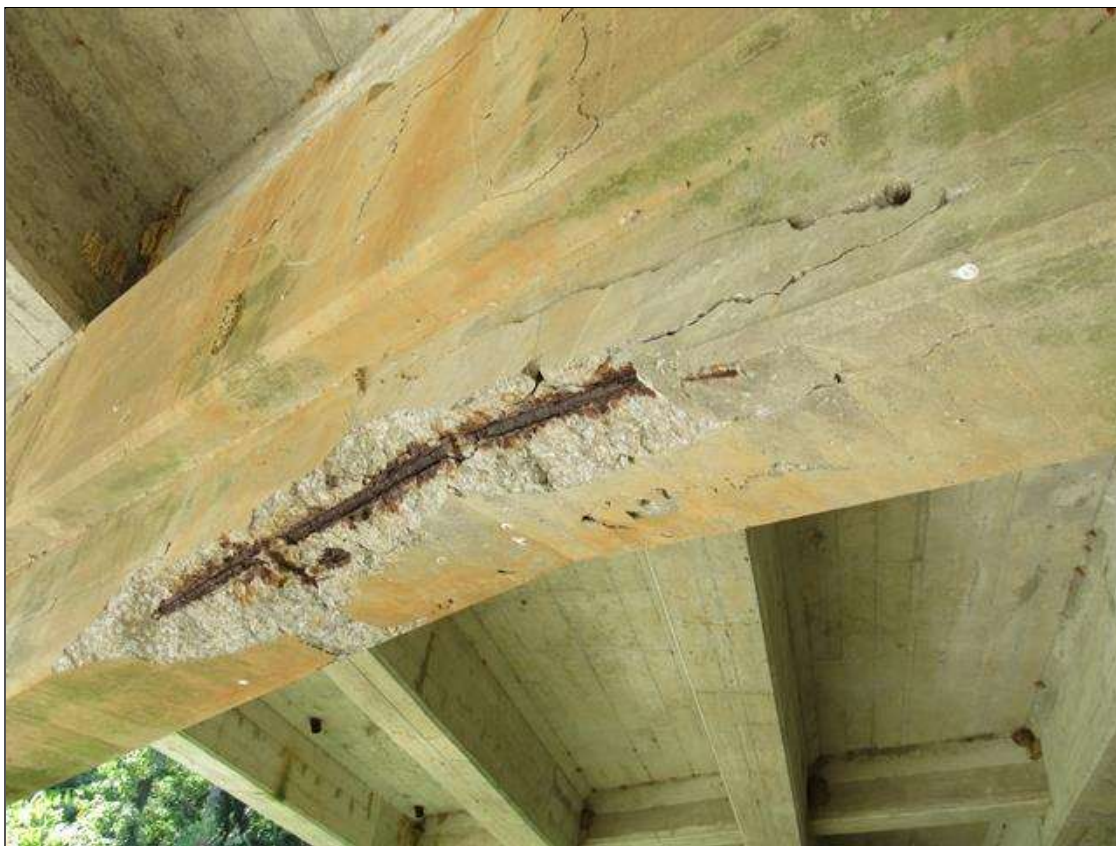
BENT 1 CAP, UNDERSIDE - SPALL/DELAM (9FT X 2FT X 5IN) WITH EXPOSED REINFORCING, UNDER BEAM 3. (PAR PHOTO)
