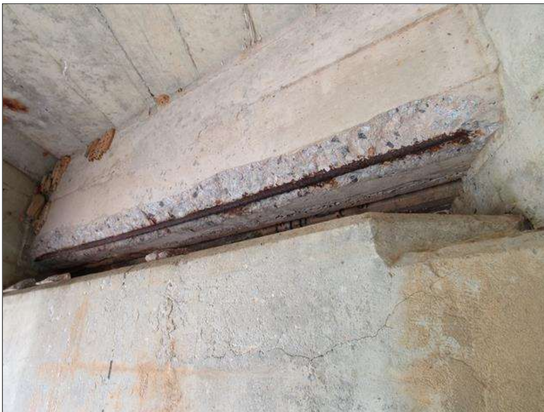
SPAN 6 NEAR END DIAPHRAGM, BAY 4 - SPALL (5FT X 6IN X 3IN) WITH EXPOSED REINFORCING
