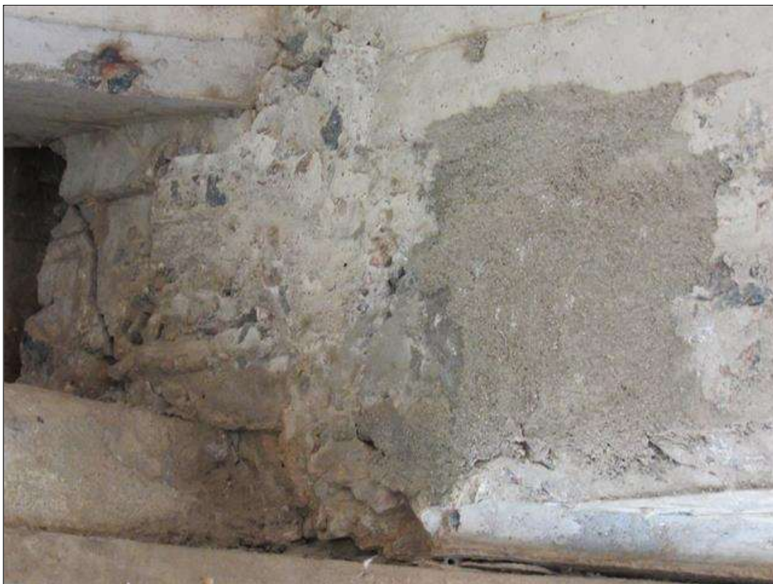
SPAN 1 BEAM 4 - SOUND PATCH (8IN DIAM) & DIAGONAL OPEN CRACK, (UP TO 1/8IN X 5IN L.) LEFT SIDE AT FAR END
