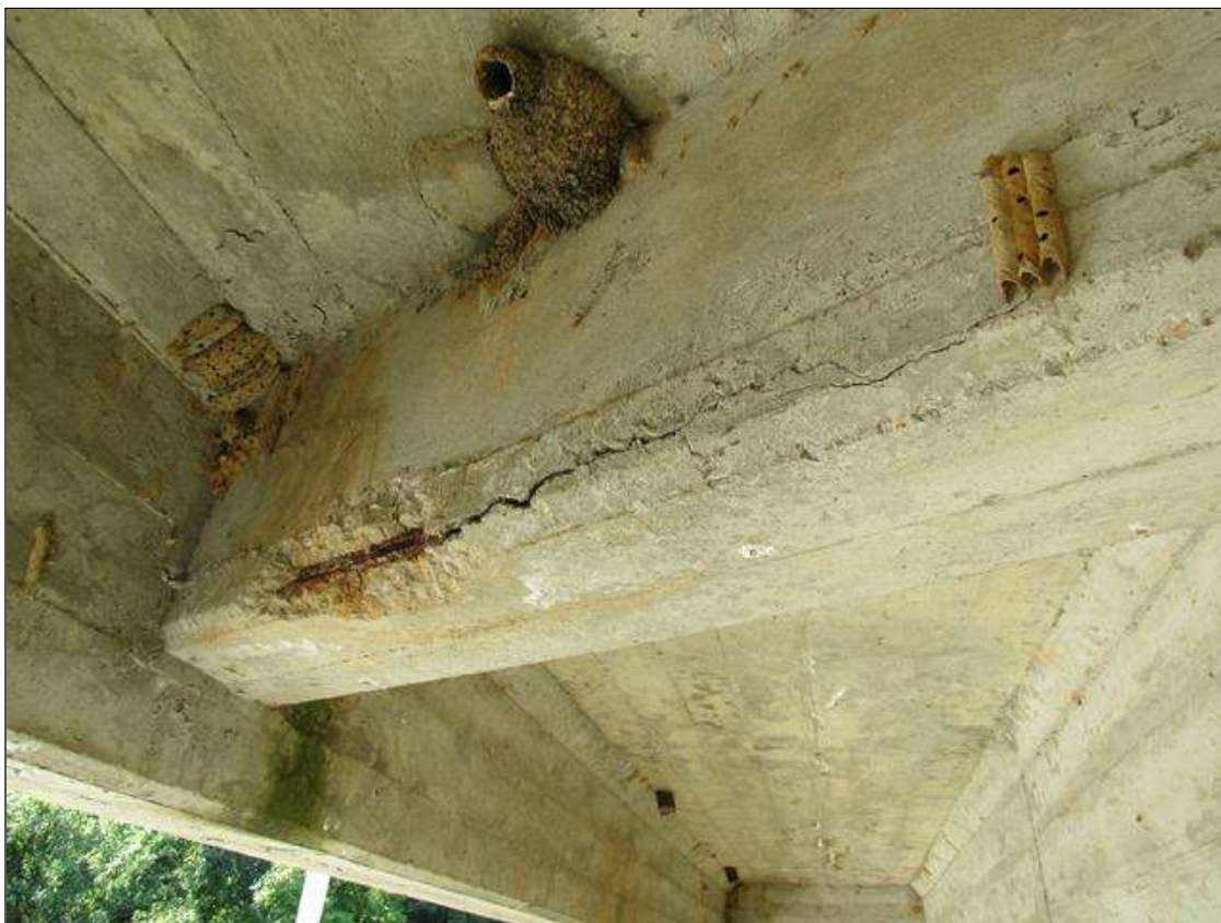
SPAN 2 BAY 4 MID-SPAN DIAPHRAGM - SPALL/DELAM (3FT X 6IN X 3IN) WITH REINFORCING EXPOSED
