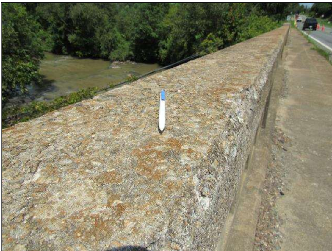
TYPICAL WEAR WITH EXPOSED AGGREGATE THROUGHOUT TOP OF RAIL, SPAN 3 LEFT RAIL
