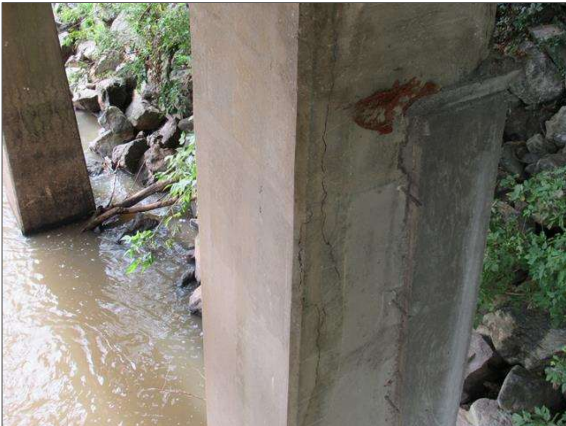
BENT 1 COLUMN 1 - DELAM (6FT X 8IN ) FAR LEFT CORNER, STARTING 2FT FROM BOTTOM OF CAP
