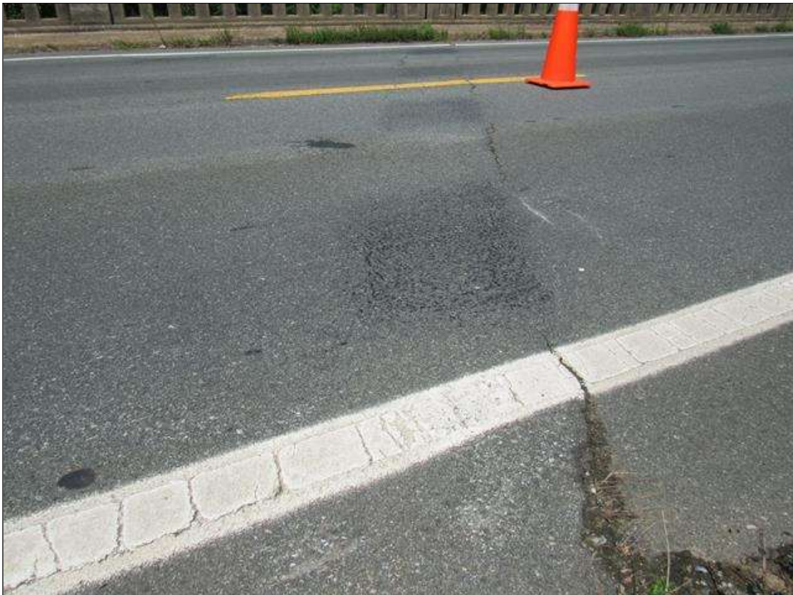
TYPICAL AWS OVER INTERIOR BENT - TRANSVERSE OPEN CRACKING, (UP TO 1/4IN X FULL W.) THROUGHOUT, AWS OVER BENT 3
