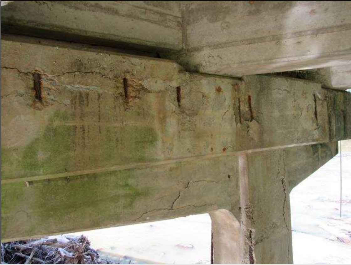
BENT 4 CAP, FAR FACE - INTERMITTENT SPALLING/DELAM, (UP TO 2SF X 2IN D.) WITH EXPOSED REINFORCING, BETWEEN BEAMS 1 & 3
