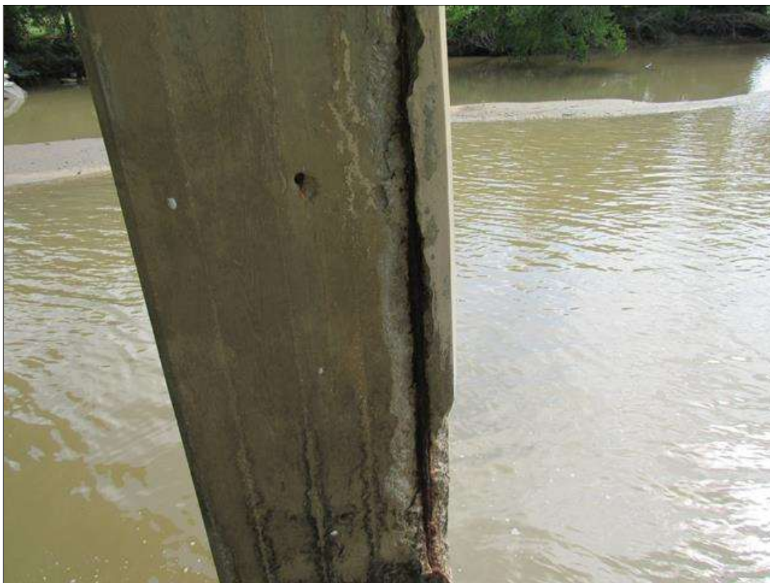
BENT 2 COLUMN 2 - SPALL/DELAM (10FT X 1FT X 4IN) WITH EXPOSED REINFORCING, NEAR RIGHT CORNER, STARTING 6FT DOWN FROM CAP. (PAR PHOTO)
