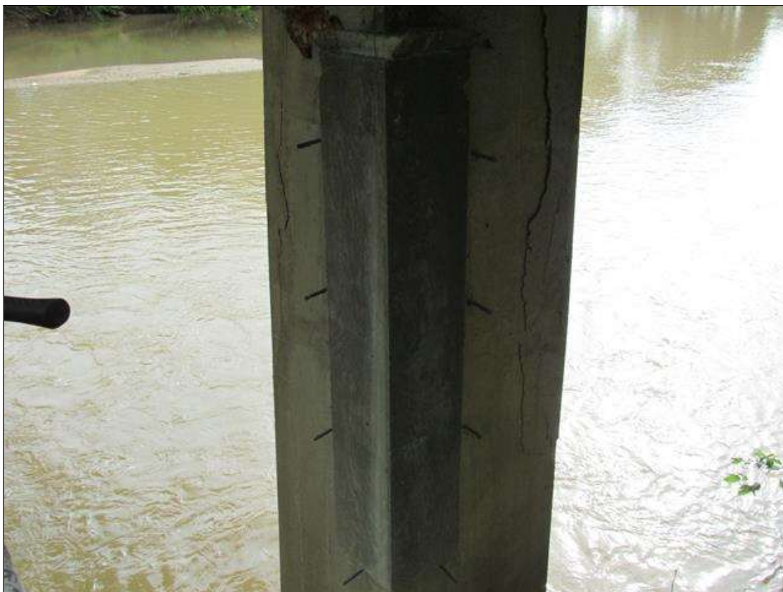
BENT 1 COLUMN 1 - SOUND PATCH (6FT X 2FT) NEAR LEFT CORNER, 3FT FROM BOTTOM OF CAP
