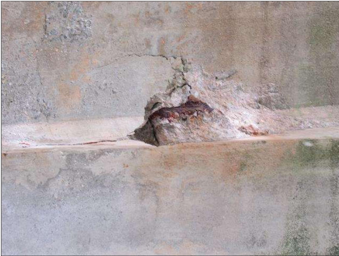
BENT 4 CAP, FAR FACE - SPALL (2FT X 8IN X 4IN) WITH EXPOSED REINFORCING, UNDER BEAM 4
