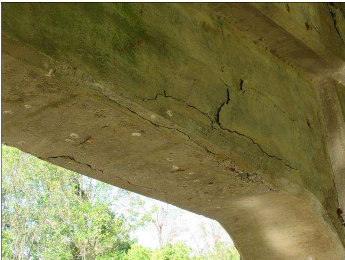
BENT 4 CAP, FAR FACE - DELAM (4FT X FULL W.) TO GUSSET UNDER BEAM 2
