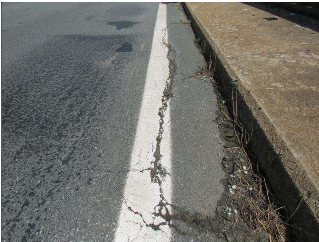
TYPICAL INTERMITTENT LONGITUDINAL OPEN CRACKING, (UP TO 1/2IN X 8FTL.) THROUGHOUT, SPAN 2 NEAR END RIGHT SIDE
