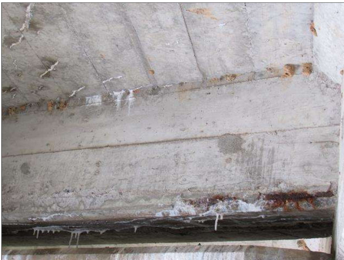
SPAN 3 NEAR END DIAPHRAGM, BAY 1 - SPALL (2FT X 4IN X 1IN) WITH EXPOSED REINFORCING & EFFLO.
