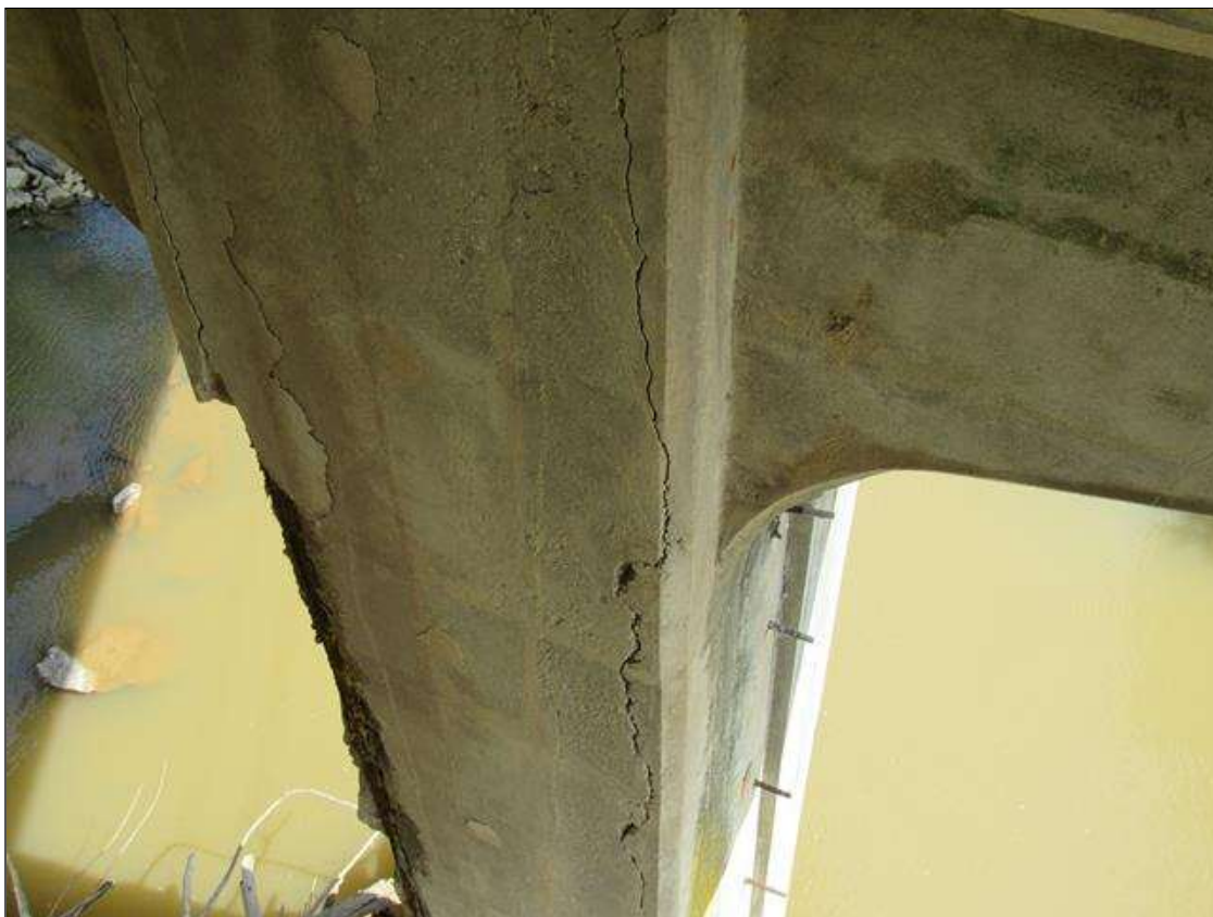
BENT 4 COLUMN 1 - DELAM (8FT X 10IN) NEAR RIGHT CORNER STARTING AT CAP
