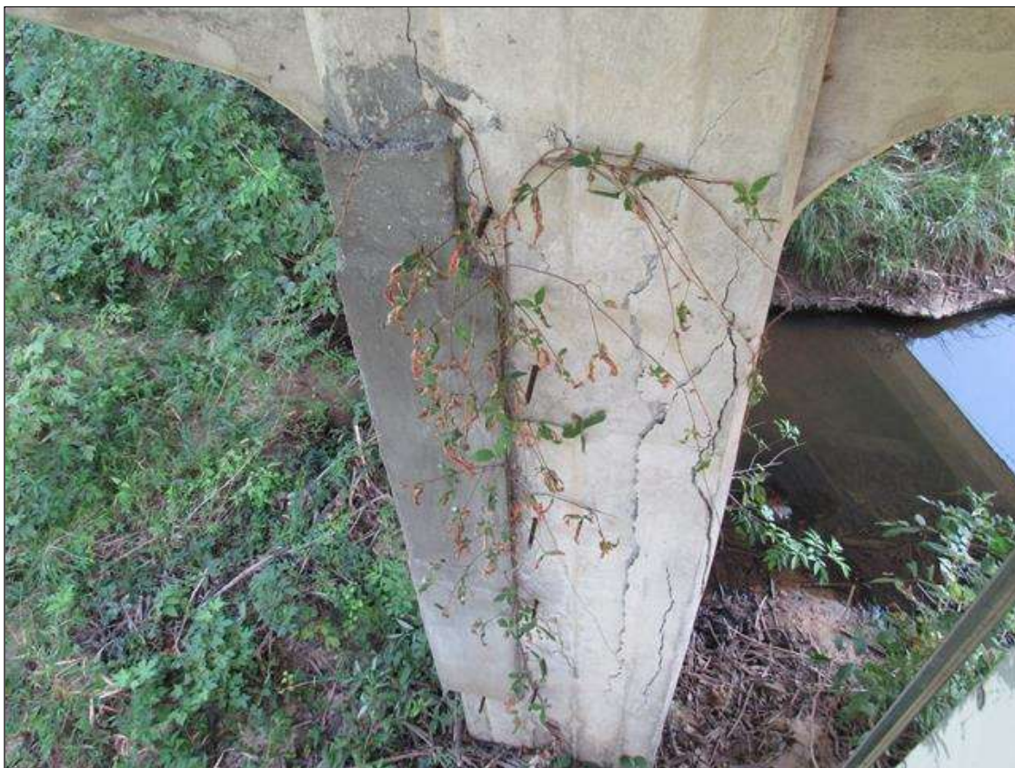
BENT 5 COLUMN 1 - PRATIALLY DELAMINATED PATCH, (1SF) AT TOP TO NEAR LEFT CORNER & DELAM (10FT X 1FT) TO NEAR RIGHT CORNER
