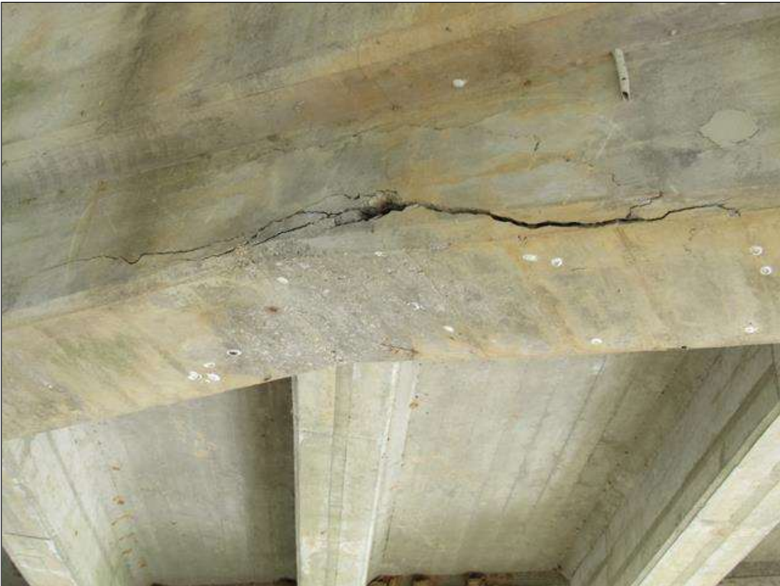
BENT 4 CAP NEAR FACE - DELAM/SPALL (4SF X 3IN D.) WITH EXPOSED REINFORCING, UNDER BEAM 3 TO GUSSET
