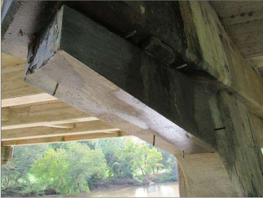
BENT 1 NEAR FACE - PARTIALLY DELAMINATED PATCH, (1SF) AT LEFT END
