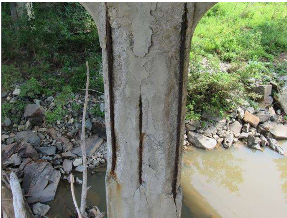
BENT 4 COLUMN 1 - SPALL/DELAM (13FT L. X FULL W. X 6IN D.) WITH EXPOSED REINFORCING, NEAR FACE. (PAR PHOTO)
