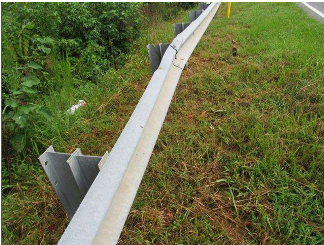
FAR LEFT GUARDRAIL - MODERATE DAMAGE (30FT), STARTING 50 FT FROM BRIDGE
