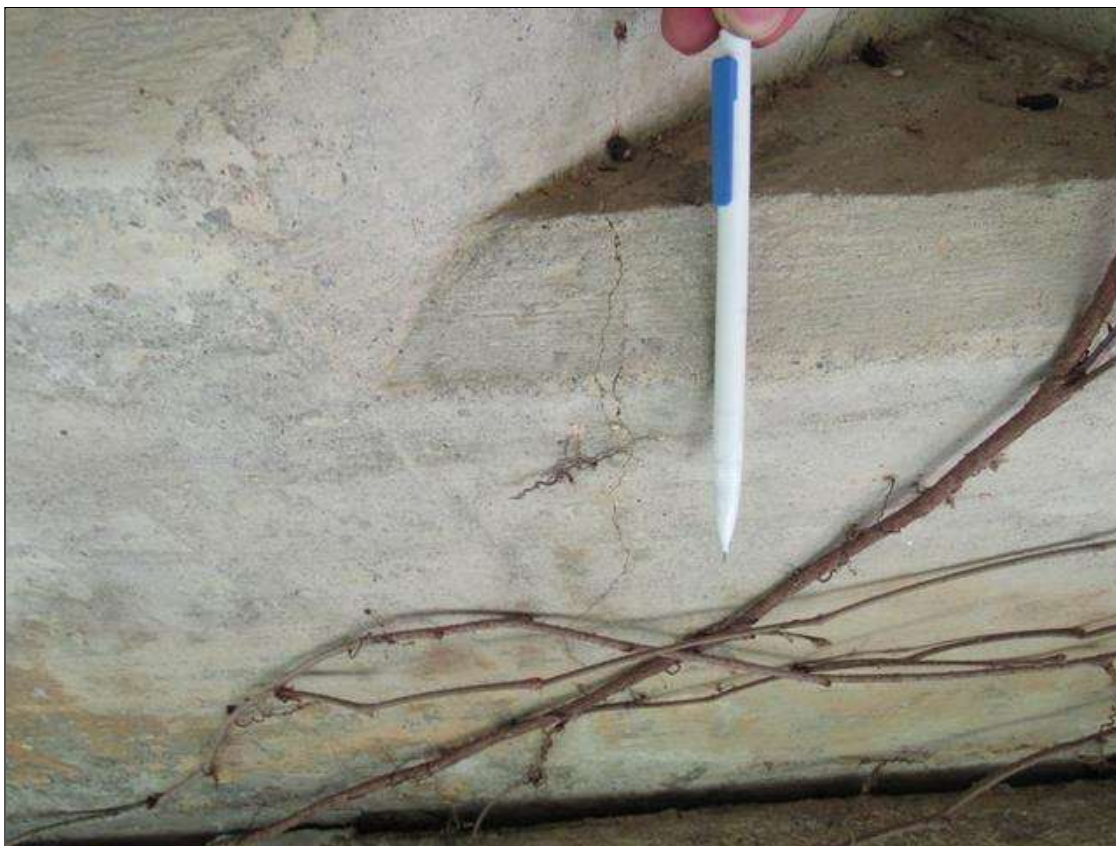
TYPICAL INTERMITTENT VERTICAL HAIRLINE CRACK, (UP TO 10IN L.) THROUGHOUT CAP, END BENT 2 BAY 1
