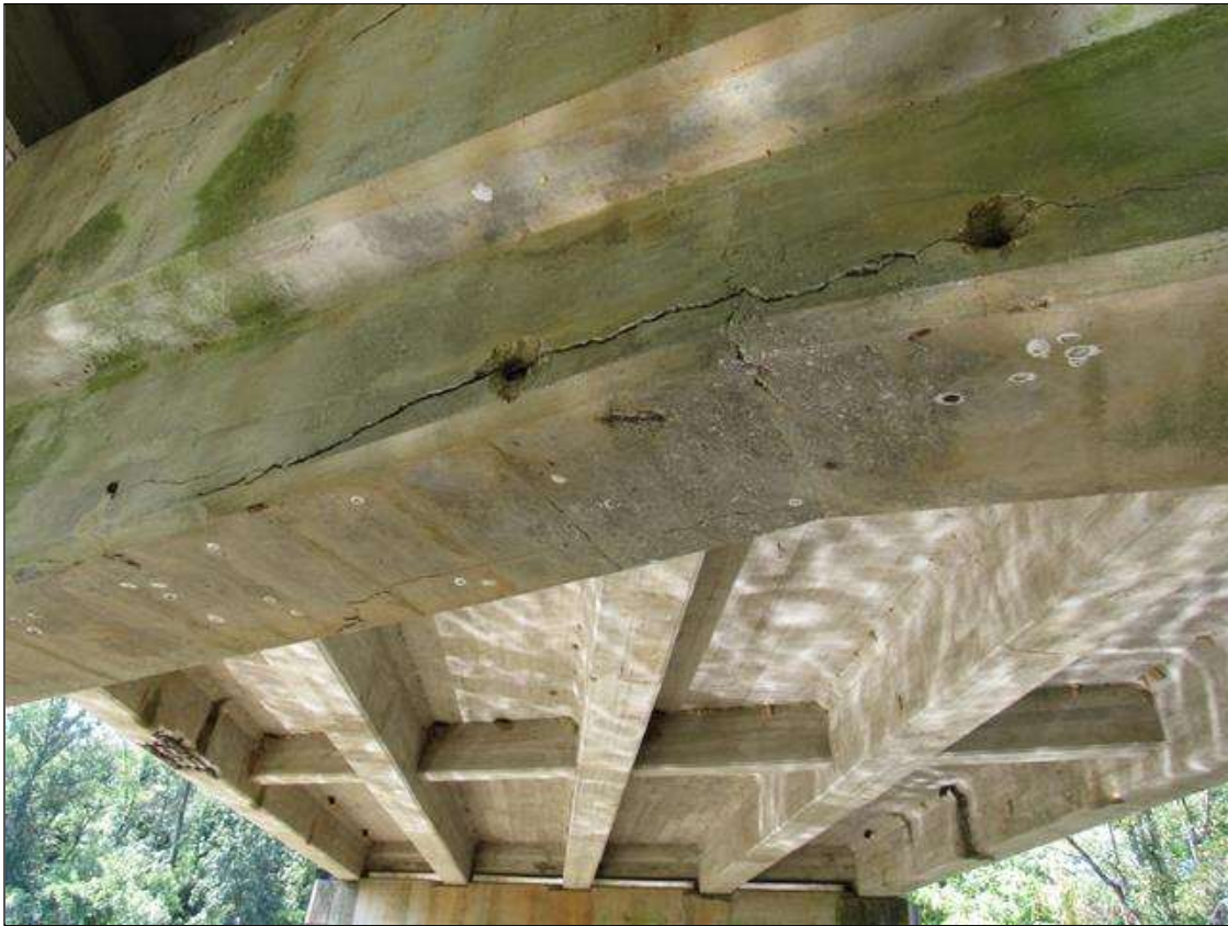
BENT 4 CAP, FAR FACE - DELAM (5FT X FULL W.) TO BOTTOM UNDER BEAM 3
