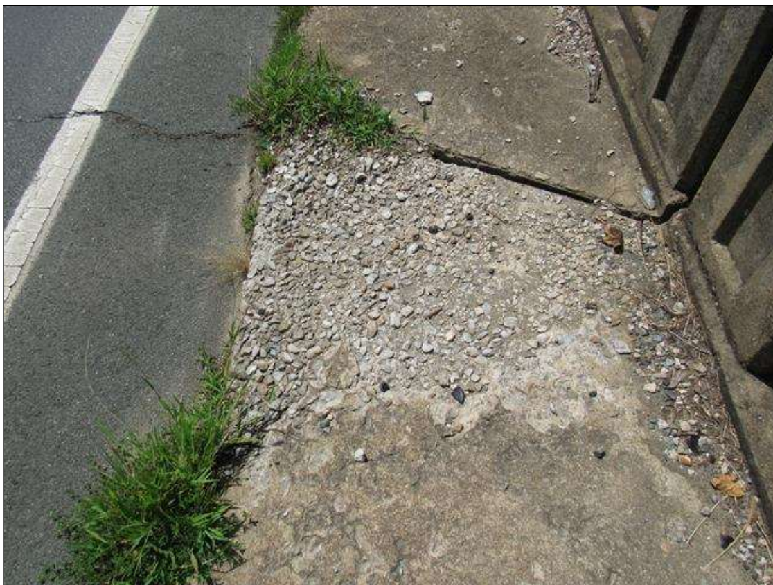
SPAN 3 SIDEWALK, LEFT SIDE - SPALLING, (4FT X 4FT X 3IN) WITH EXPOSED REINFORCING & LOOSE AGGREGATE, NEAR END. (PAR PHOTO)
