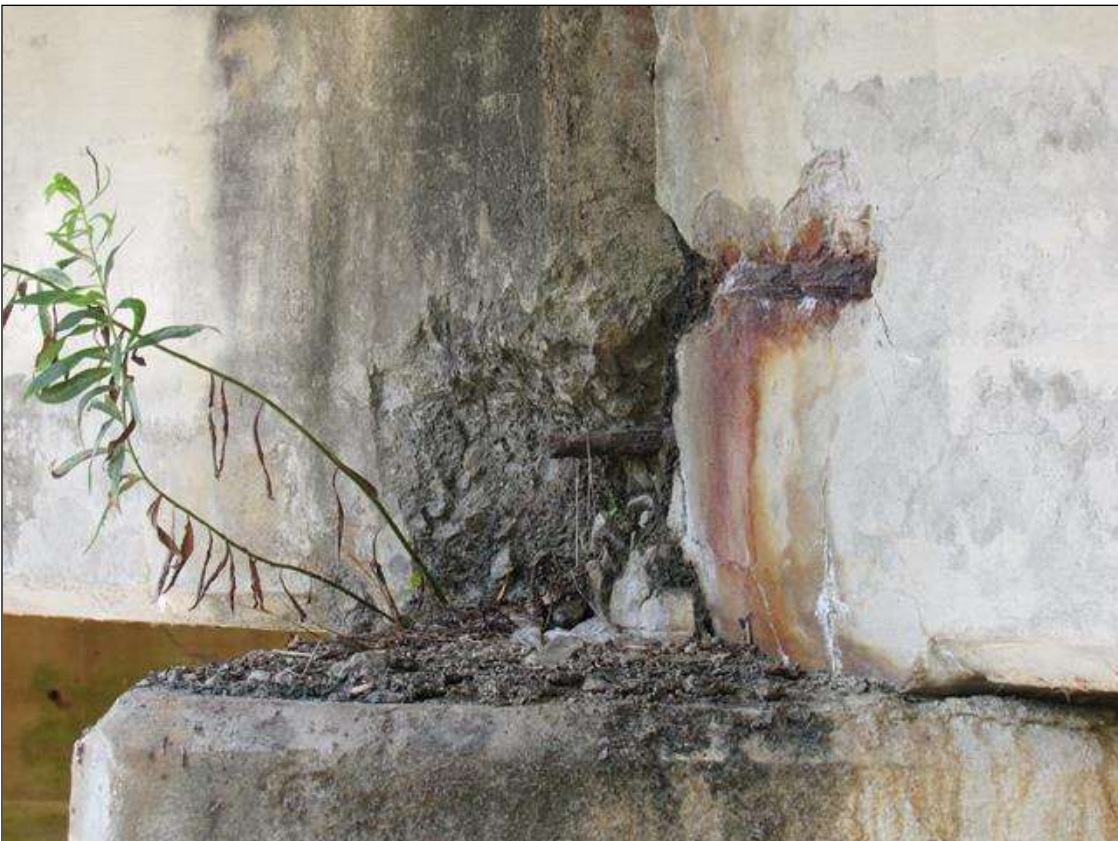
SPAN 4 FAR END, SPAN 5 NEAR END, BEAM 5 - SPALL/DELAM (UP TO 1SF X 4IN D.) WITH EXPOSED REINFORCING & BEARING LOSS TO SPAN 4 BEAM 5 ONLY (12IN X 4IN), RIGHT SIDE FAR END. (PAR PHOTO)
