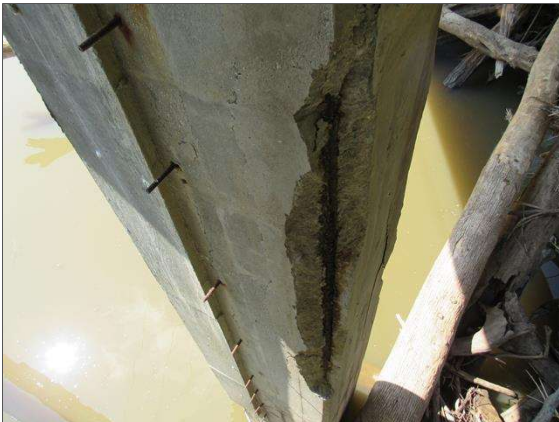
BENT 4 COLUMN 2 - SPALL/DELAM (12FT L. X 1FT W. X 5IN D.) WITH EXPOSED REINFORCING, FAR LEFT CORNER. (PAR PHOTO)
