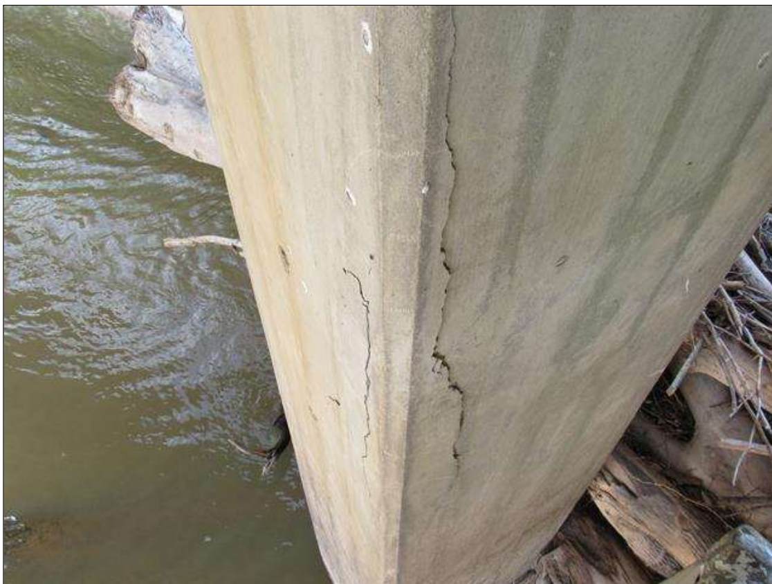
BENT 3 COLUMN 1 - DELAM (5FT X 8IN) FAR RIGHT CORNER STARTING 5FT FROM CAP
