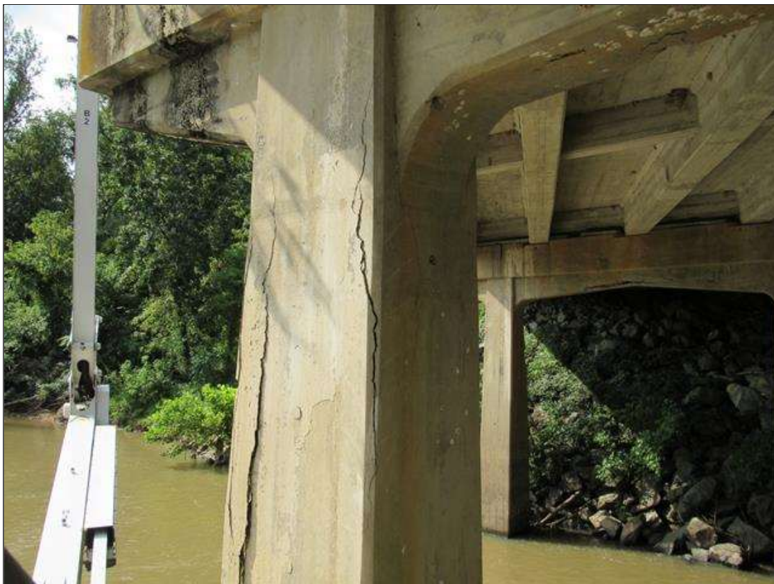
BENT 2 COLUMN 2 - DELAM (6FT X 1FT) FAR LEFT CORNER STARTING AT CAP
