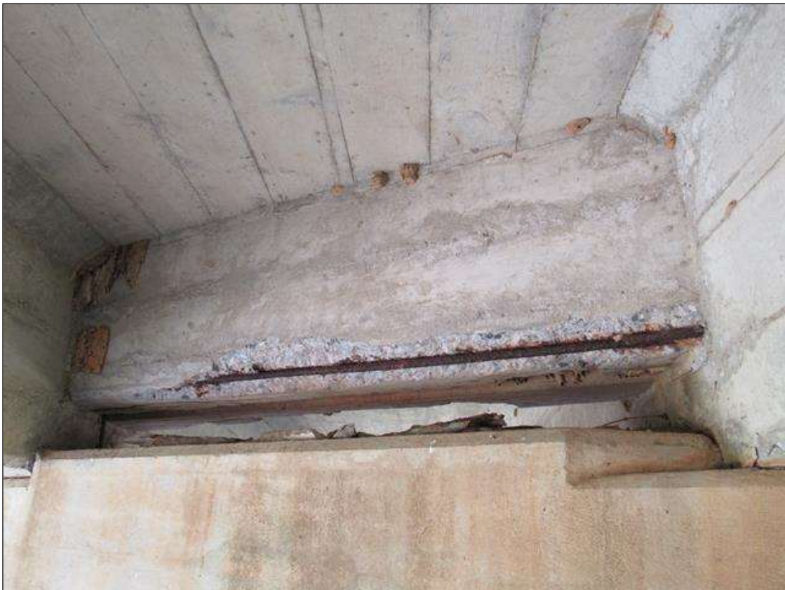
SPAN 6 NEAR END DIAPHRAGM, BAY 3 - SPALL (4FT X 6IN X 3IN) WITH EXPOSED REINFORCING
