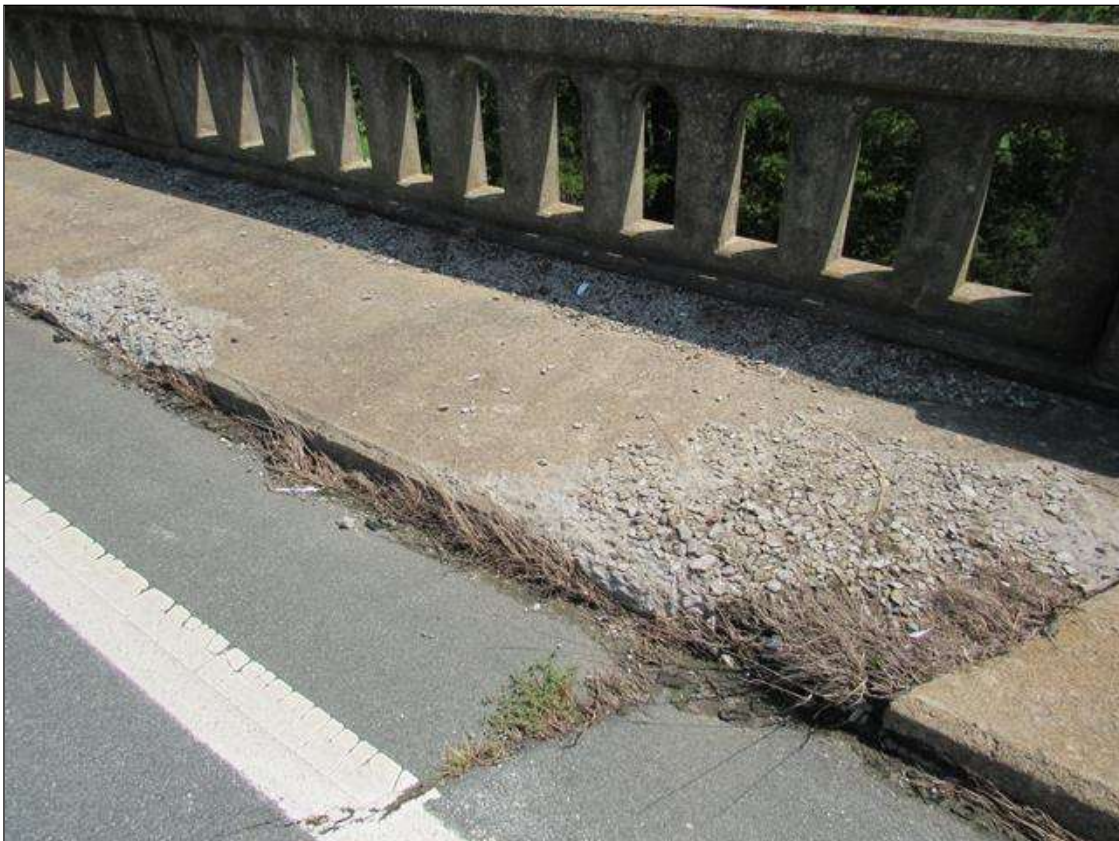
SPAN 5 SIDEWALK, RIGHT SIDE - SPALLING, (UP TO 5FT X 4FT X 3IN) WITH EXPOSED REINFORCING & LOOSE AGGREGATE, NEAR END. (PAR PHOTO)
