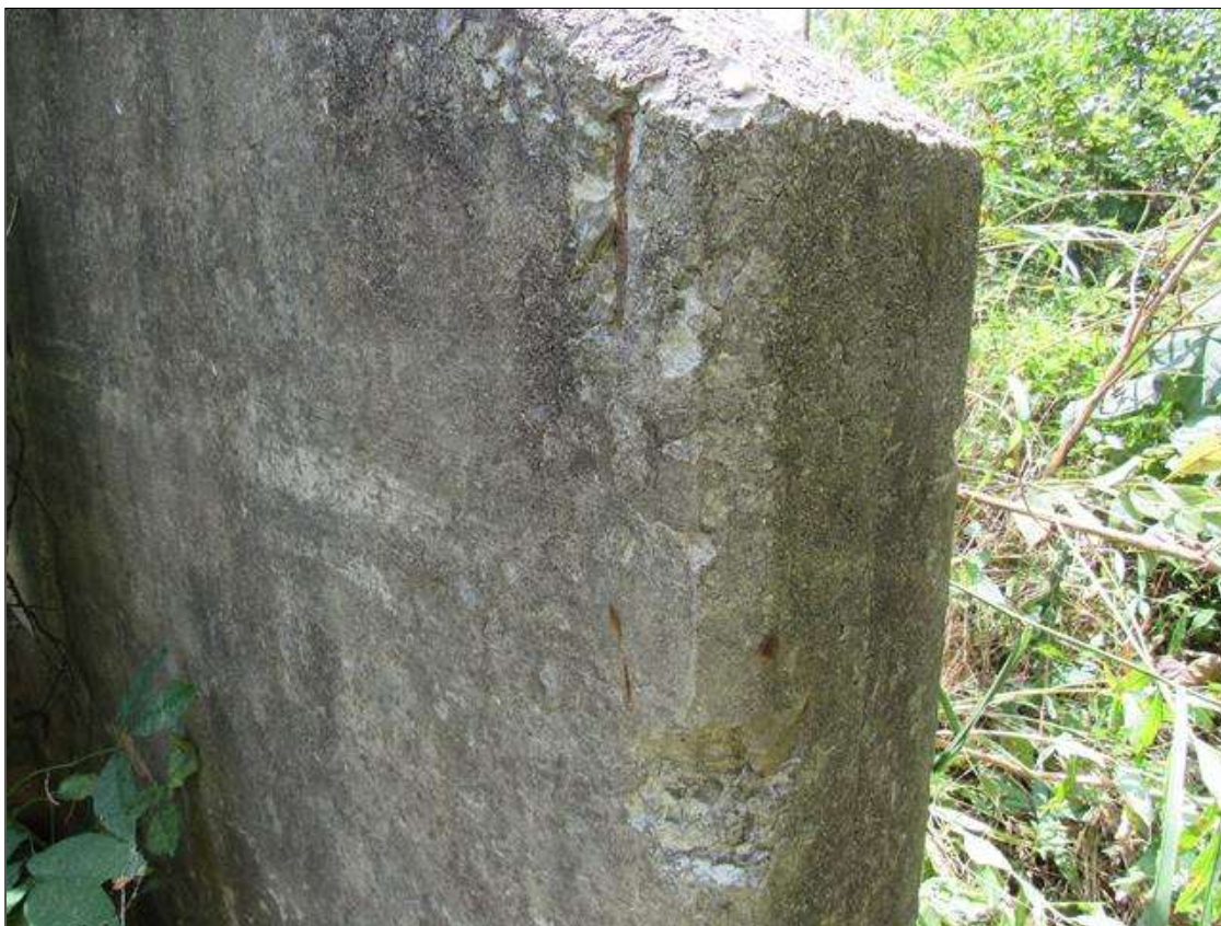
NEAR LEFT WINGWALL - SPALLING, (UP TO 6IN X 4IN X 1/2IN) WITH EXPOSED REINFORCING, FAR CORNER
