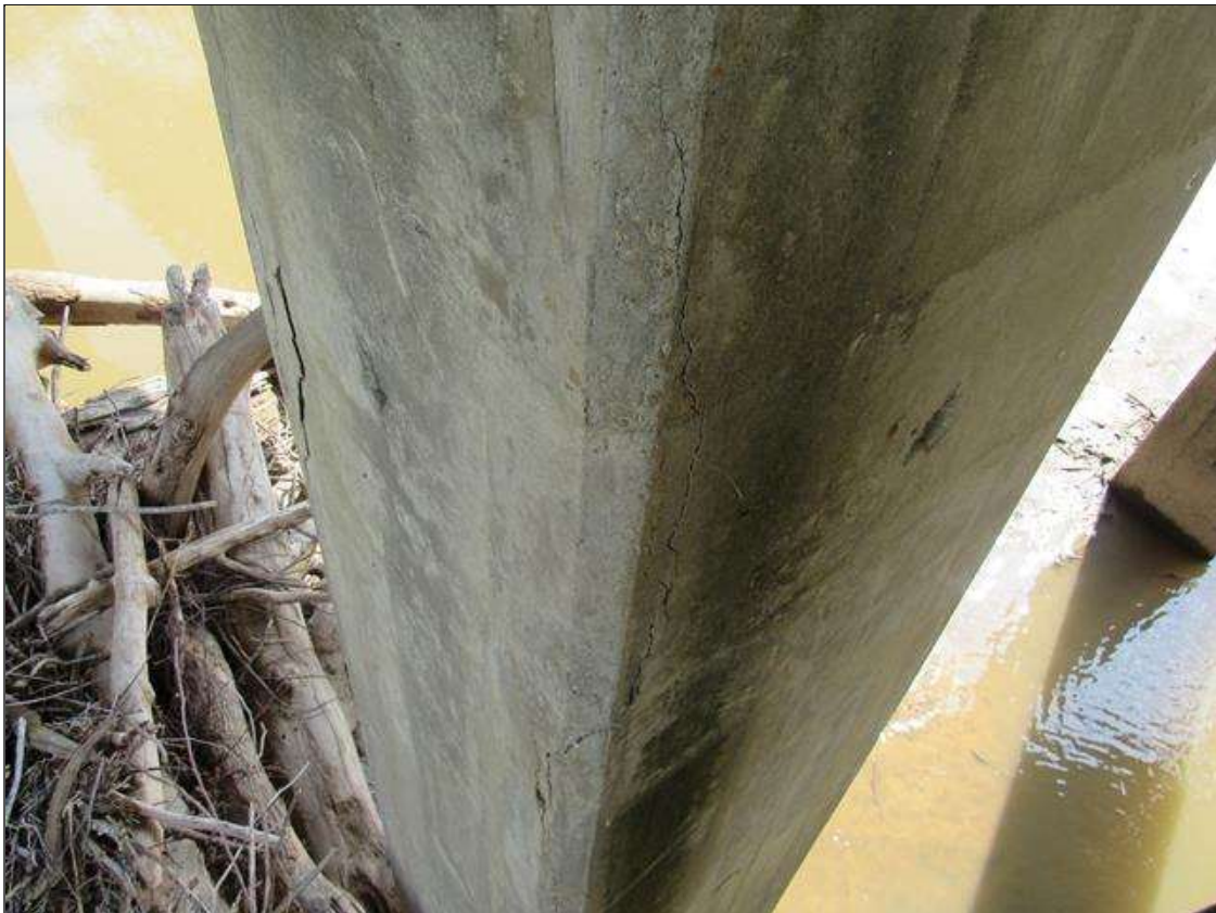
BENT 3 COLUMN 1 - DELAM (2.5FT X 6IN) NEAR LEFT CORNER, STARTING 2FT FROM CAP
