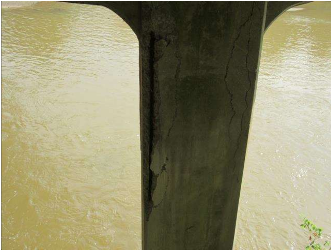
BENT 1 COLUMN 2 - SPALL/DELAM (7FT X 1FT X 4IN) WITH EXPOSED REINFORCING, NEAR LEFT CORNER STARTING AT TOP OF COLUMN. (PAR PHOTO)
