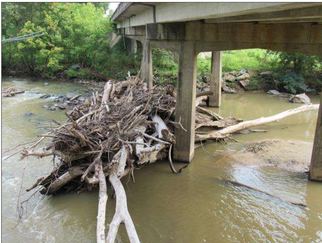
DRIFT, (100FT L. X 50FT W. X 15FT D.) UPSTREAM SIDE SPAN 4. (PAR PHOTO)
