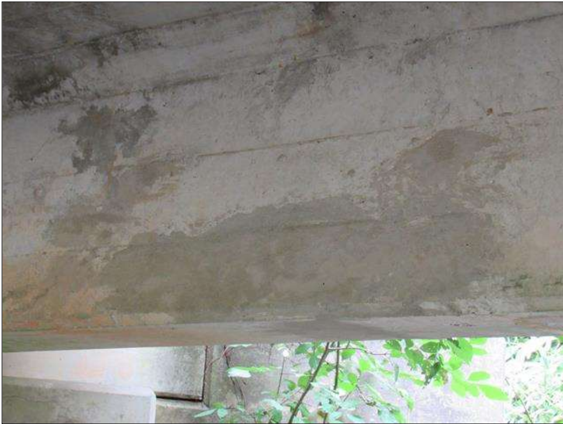
TYPICAL INTERMITTENT SOUND PATCH, (UP TO 3SF) THROUGHOUT BEAMS, SPAN 1 BEAM 1 RIGHT SIDE, 5FT FROM NEAR END
