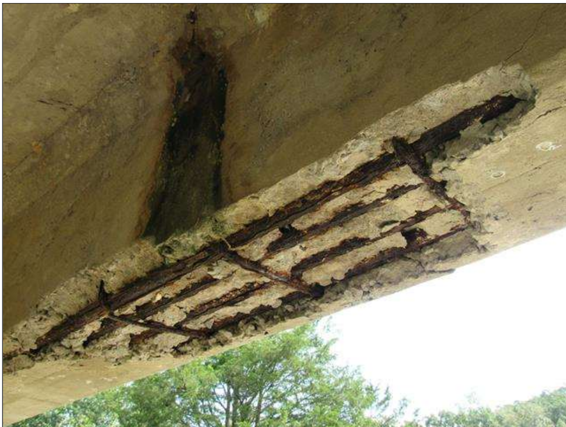
SPAN 4, BEAM 5 - SPALL (5FT X FULL W. X 5IN D.) WITH EXPOSED & CORRODED REINFORCING, BOTTOM OF BEAM AT MID-SPAN. (PAR PHOTO)
