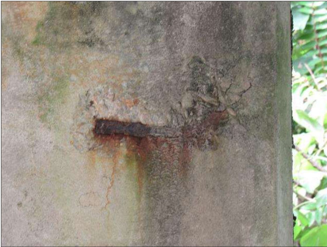
BENT 1 CAP, FAR FACE - SPALL (1FT X 6IN X 1IN) WITH EXPOSED REINFORCING, UNDER BEAM 1
