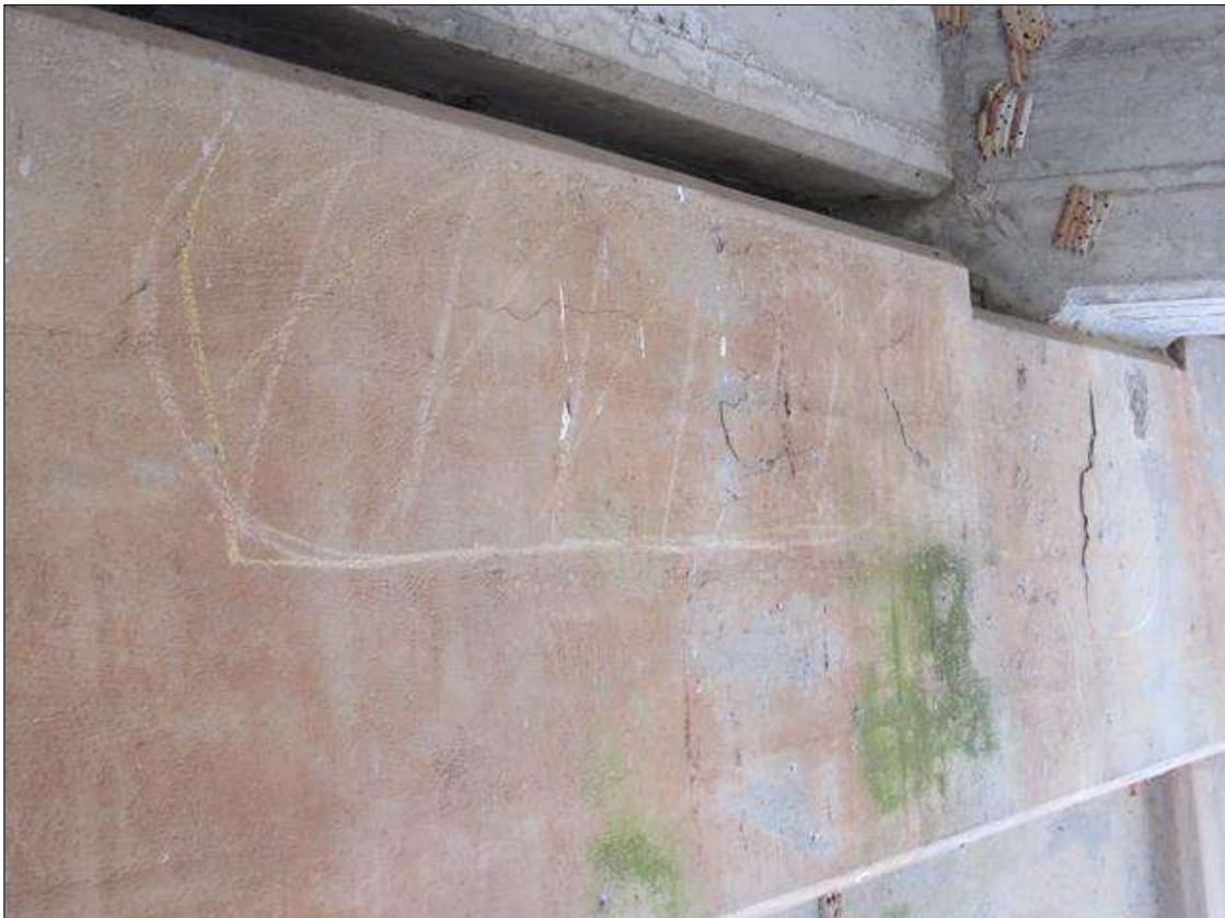
BENT 2 CAP, NEAR FACE - DELAM (5SF) UNDER BAY 3
