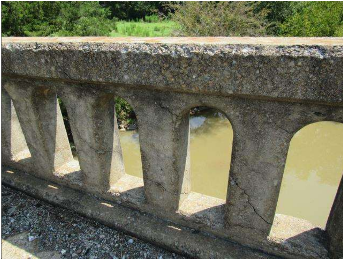
SPAN 4 RIGHT RAIL - DIAGONAL OPEN CRACKING, (UP TO 1/8IN X 4FT L.) AT 1/3 POINT
