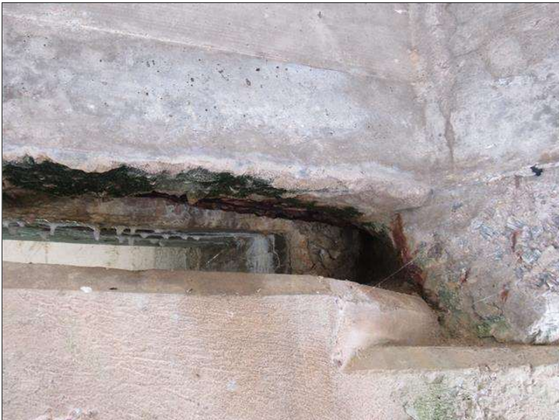
SPAN 4 BEAM 5 - SPALL (2FT X 6IN X 4IN) WITH EXPOSED REINFORCING, FAR END LEFT SIDE
