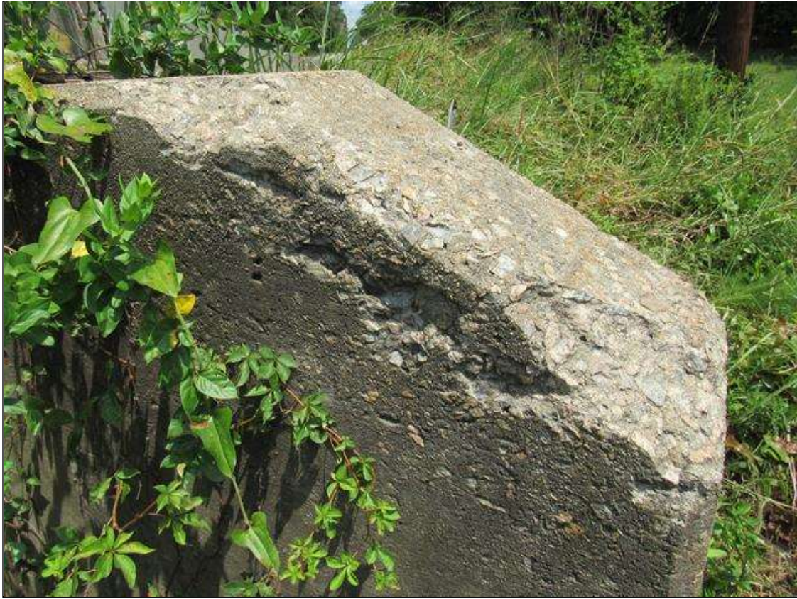
FAR RIGHT WINGWALL - SPALLING, (UP TO 2FT X 8IN X 2IN) NO EXPOSED REINFORCING, NEAR CORNER
