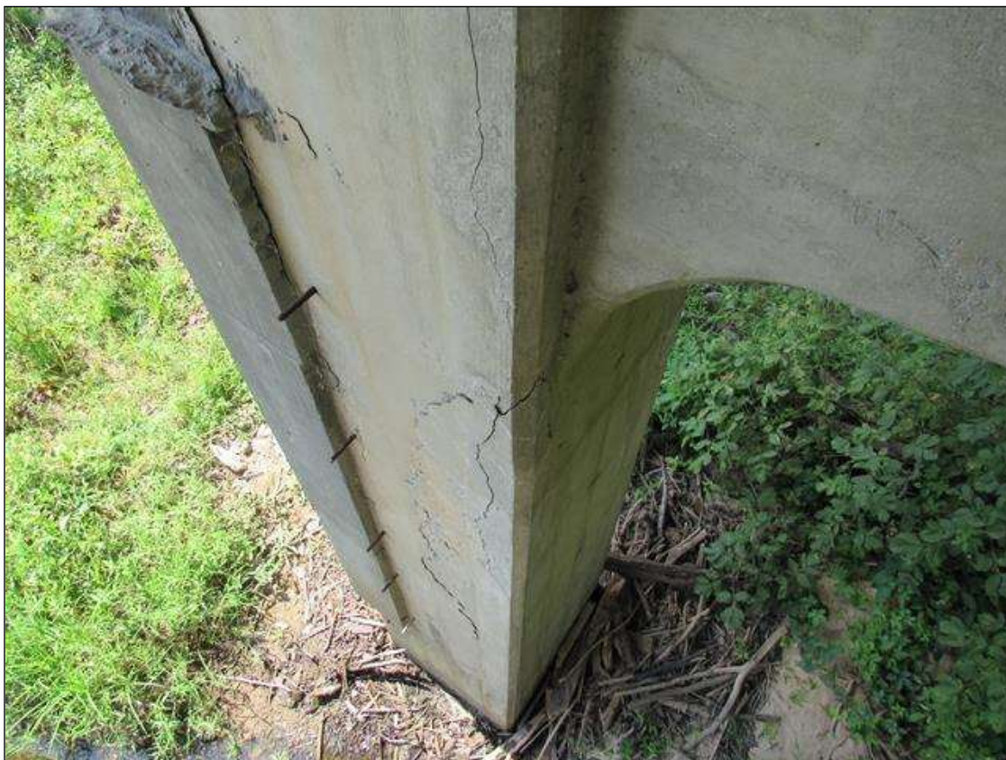
BENT 5 COLUMN 2 - DELAM (10FT X 16IN) FAR LEFT CORNER STARTING AT BOTTOM OF CAP
