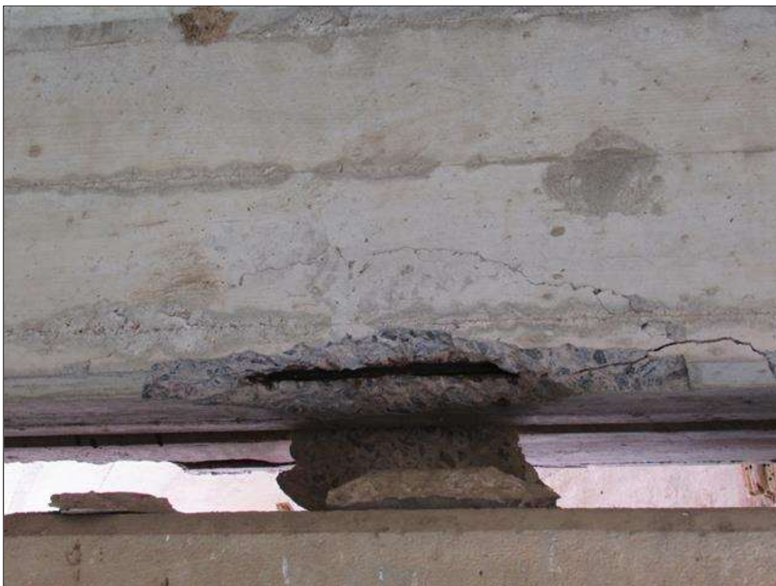
SPAN 1 FAR END DIAPHRAGM - SPALL/DELAM (3FT X 1FT X 3IN) WITH EXPOSED REBAR, LEFT OF BEAM 4
