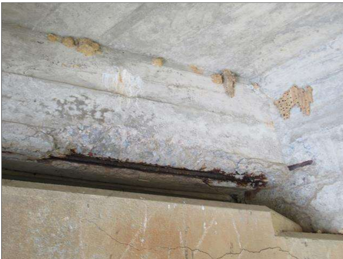
SPAN 2 NEAR END DIAPHRAGM - SPALL (3FT X 6IN X 3IN) WITH EXPOSED REINFORCING, RIGHT OF BEAM 3
