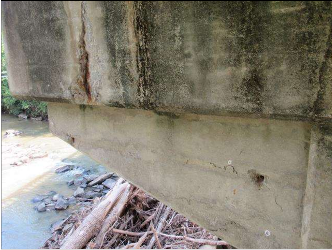
BENT 3 NEAR FACE - SPALL (18IN X 10IN X 2IN) WITH EXPOSED REINFORCING & DELAM (2SF) TO GUSSET UNDER BEAM 1
