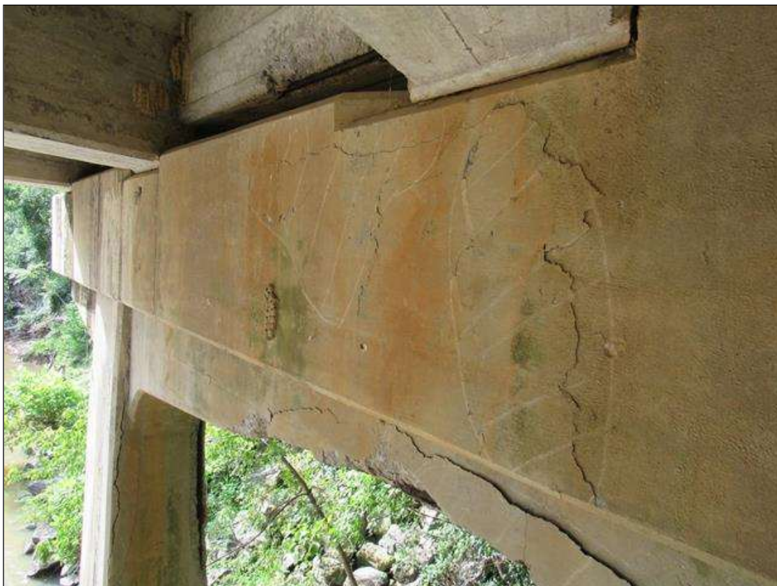
BENT 1 CAP, FAR FACE - DELAM (6SF) UNDER BEAM 3
