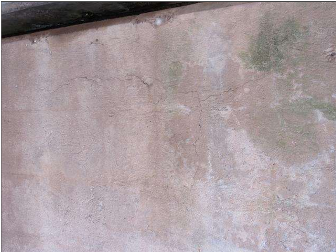
BENT 4 CAP, NEAR FACE - DELAM (1SF) ABOVE COLUMN 2
