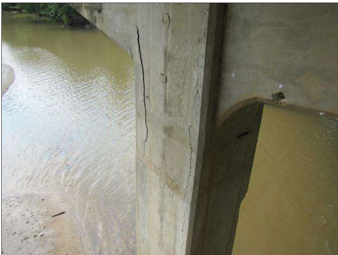
BENT 3 COLUMN 2 - (X2) DELAM (UP TO 7FT X 8IN) FAR LEFT & FAR RIGHT CORNERS, STARTING AT CAP
