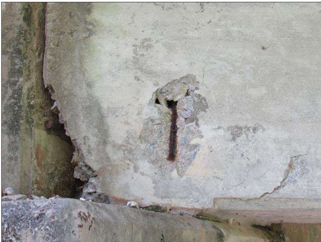
SPAN 2 BEAM 1 - SPALL/DELAM (2SF X 5IN) WITH EXPOSED REINFORCING, LEFT SIDE FAR END
