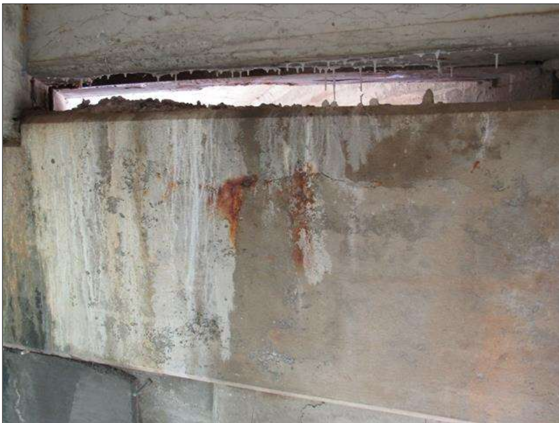
BENT 1 CAP, NEAR FACE - HORIZONTAL 1/32IN CRACK, (4FT L.) WITH EFFLO. & RUST STAINING, ABOVE COLUMN 1
