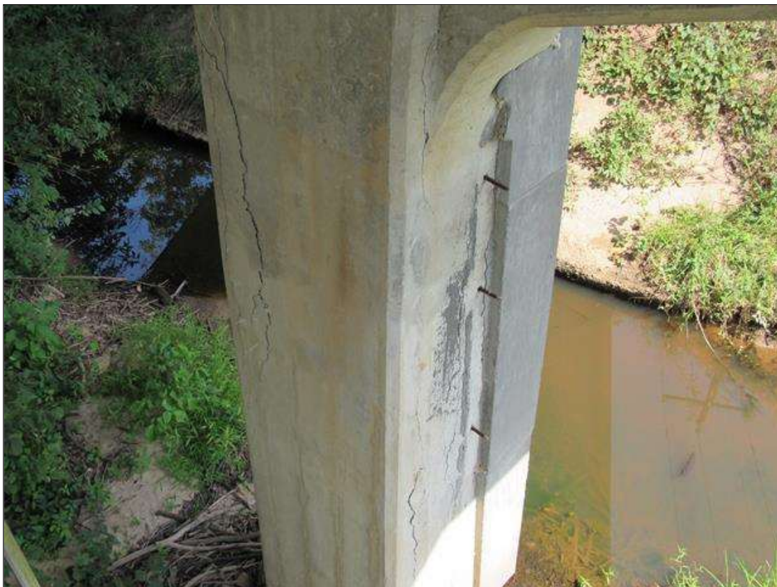
BENT 5 COLUMN 2 - DELAM (8FT X 1FT) RIGHT FACE STARTING AT TOP OF COLUMN
