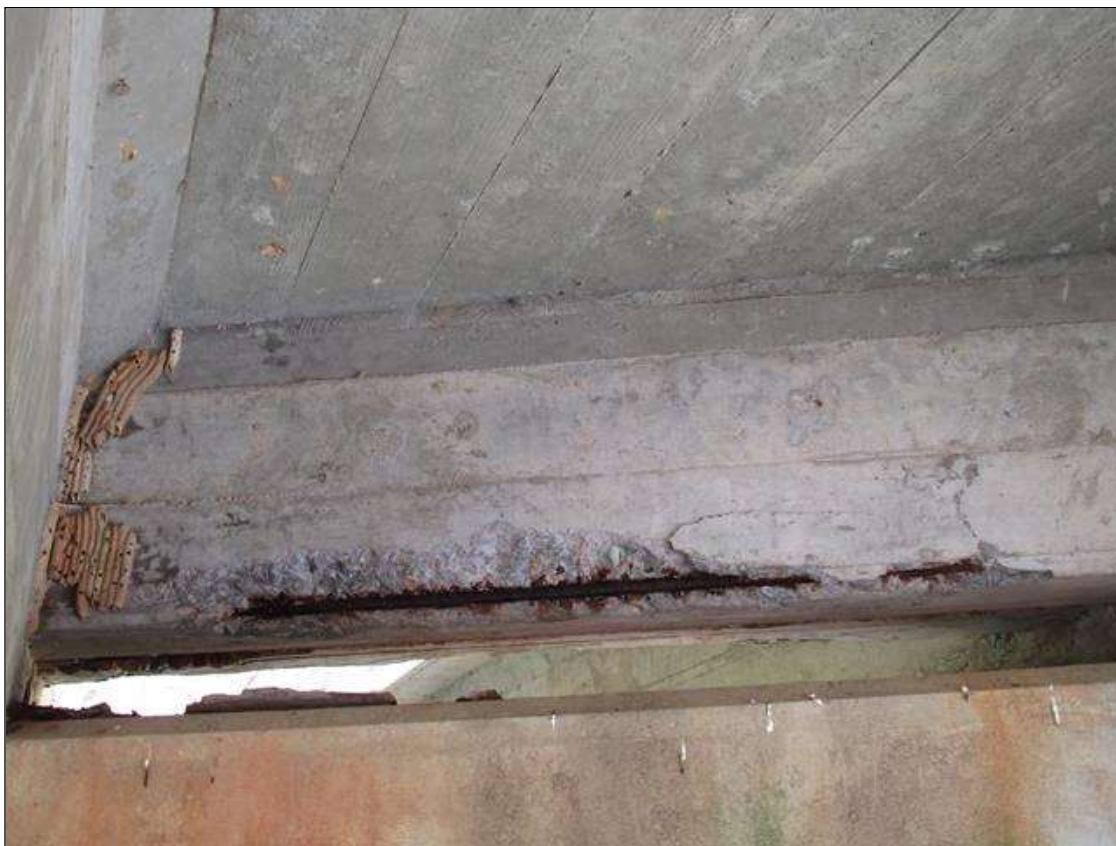
SPAN 5 FAR END DIAPHRAGM, BAY 3 - SPALL (4FT X 6IN X 3IN) WITH EXPOSED REINFORCING
