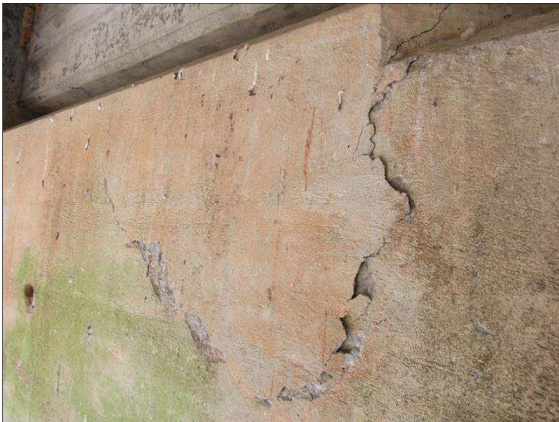
BENT 3 CAP FAR FACE - DELAM (2SF) RIGHT OF BEAM 2
