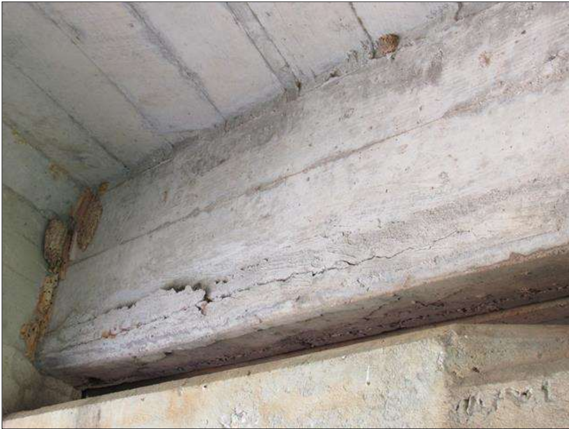
SPAN 6 NEAR END DIAPHRAGM, BAY 2 - DELAM (5FT X 6IN)
