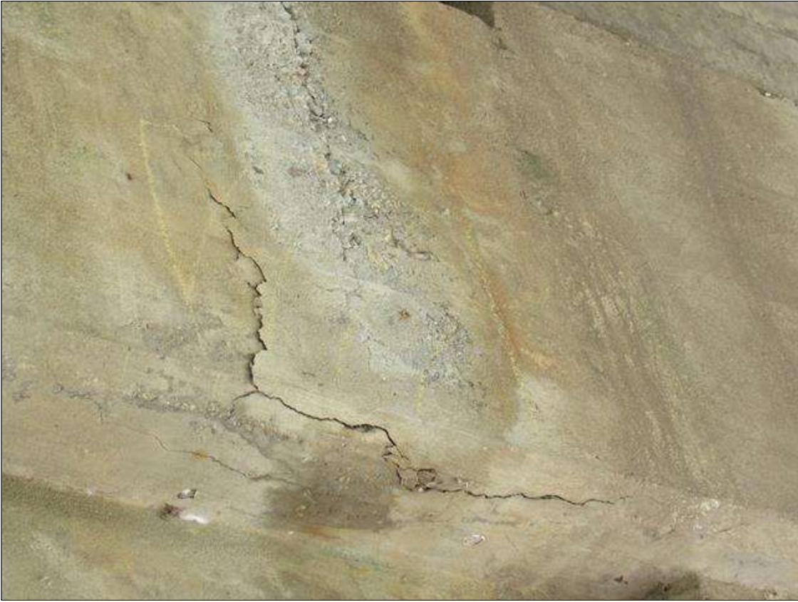
BENT 4 CAP, NEAR FACE - DELAM (1SF) UNDER BEAM 4
