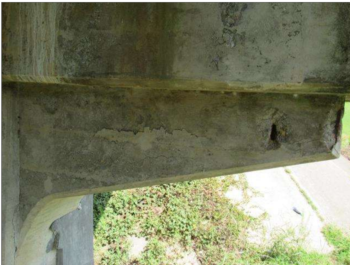
BENT 5 CAP, NEAR FACE - DELAM (2SF) & SPALLING (UP TO 6IN DIAM. X 1IN D.) WITH EXPOSED REINFORCING TO GUSSET UNDER BEAM 5
