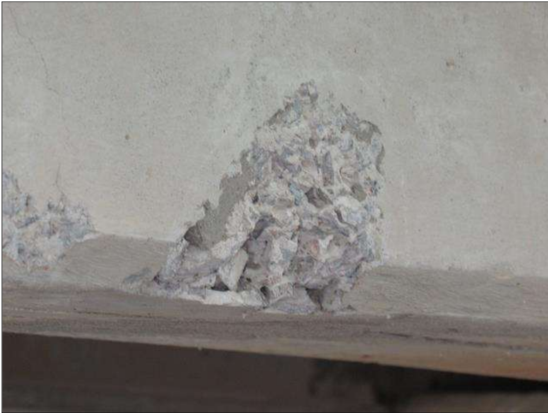
SPAN 1 BEAM 1 - SPALL (8IN X 8IN X 2IN) BOTTOM LEFT EDGE, 8FT FROM NEAR END
