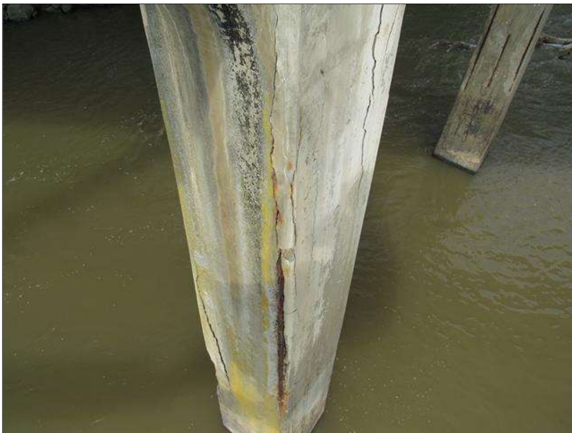
BENT 2 COLUMN 2 - SPALL/DELAM (15FT L. X 1FT W. X 6IN D.) WITH EXPOSED REINFORCING, FAR RIGHT CORNER STARTING AT CAP. (PAR PHOTO)
