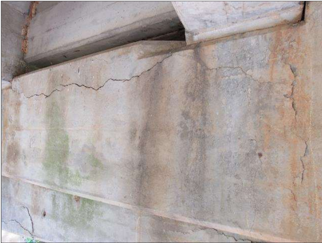
BENT 4 CAP, NEAR FACE - DELAM (UP TO 10SF) BETWEEN BEAMS 2 & 3
