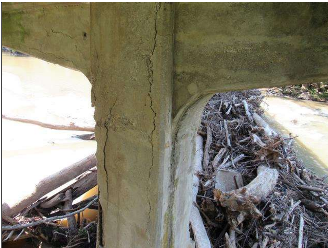
BENT 4 COLUMN 1 - DELAM (12FT X 10IN) FAR LEFT CORNER STARTING AT TOP OF COLUMN
