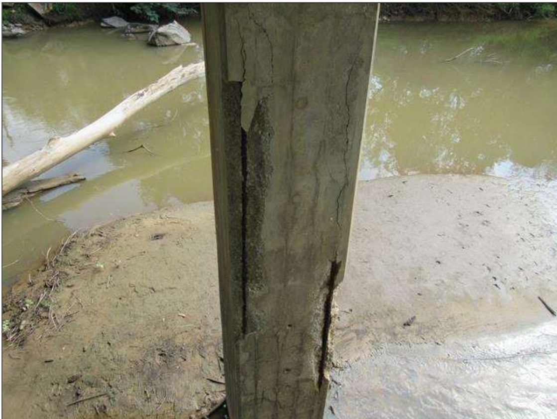
BENT 3 COLUMN 2 - (X2) SPALL/DELAM (UP TO 18FT L. X 1FT W. X 5IN D.) WITH EXPOSED REINFORCING, NEAR FACE LEFT & RIGHT CORNERS. (PAR PHOTO)
