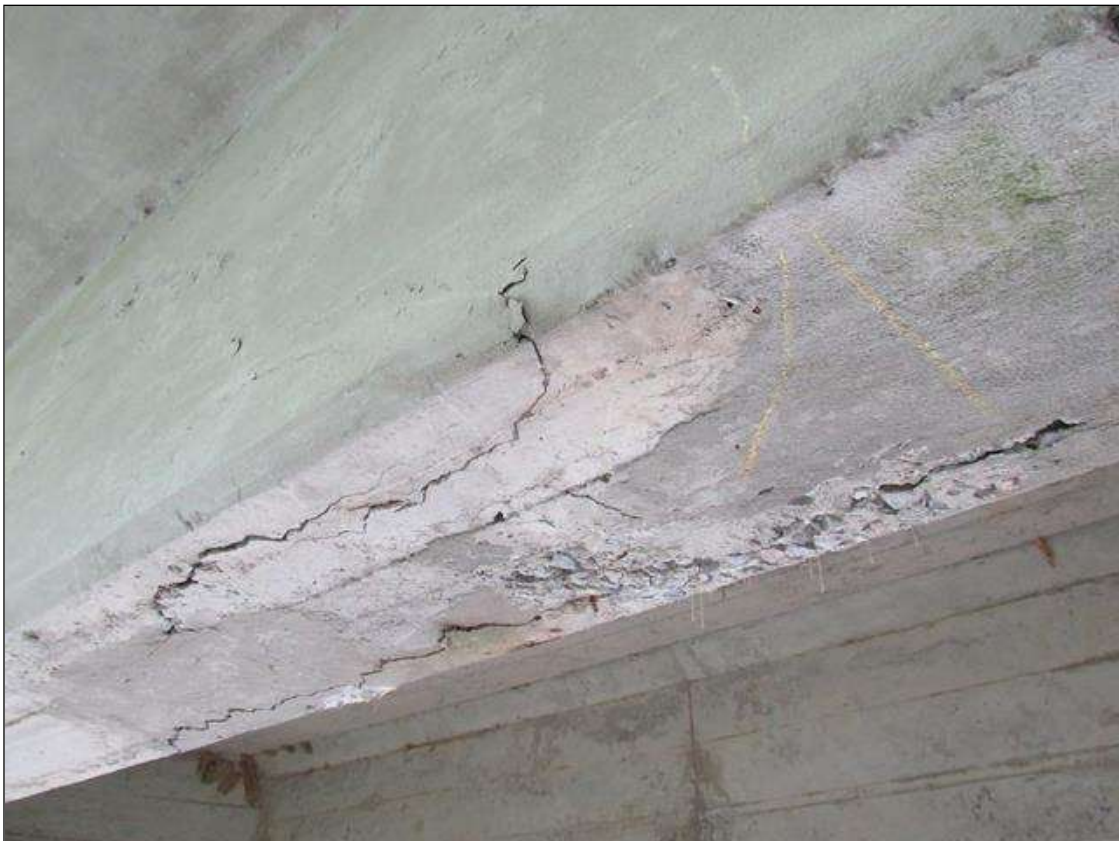
SPAN 1 BEAM 1 - DELAM (5FT L. X FULL W.) TO BOTTOM, 12FT FROM FAR END
