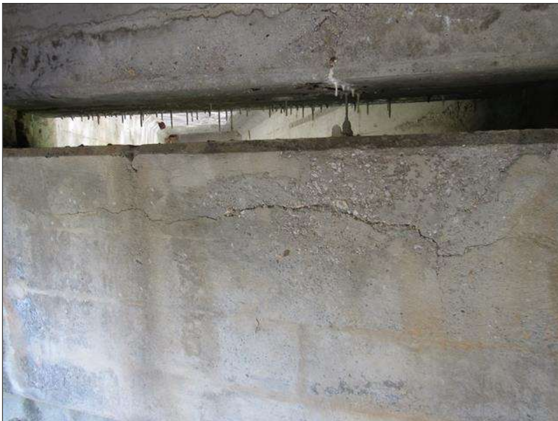
BENT 4 CAP, NEAR FACE - DELAM (5FT X 8IN) BAY 1
