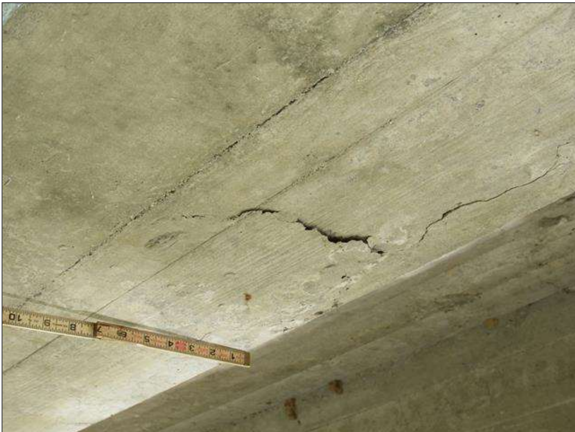
SPAN 4 BEAM 1 - DELAM (8IN DIAM.) BOTTOM OF BEAM 6FT FROM NEAR END
