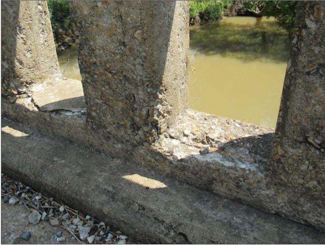
TYPICAL INTERMITTENT SPALLING, (UP TO 8IN X 2IN X 1IN) WITH EXPOSED REINFORCING & CRACKING, (UP TO 1/32IN X 2FT L.) THROUGHOUT RAIL, SPAN 3 RIGHT RAIL MID-SPAN
