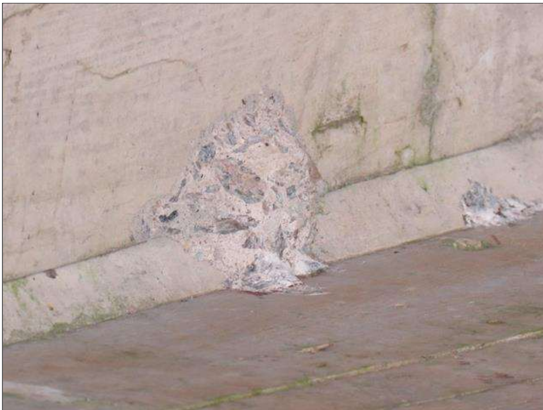
SPAN 1 BEAM 2 - SPALL (5IN X 4IN X 1IN) BOTTOM RIGHT, 10FT FROM NEAR END
