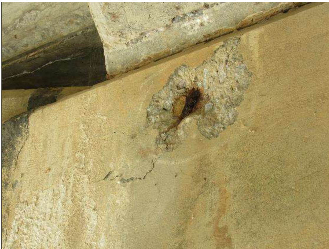
BENT 1 CAP, FAR FACE - SPALL (6IN X 1IN) WITH EXPOSED REINFORCING, UNDER BEAM 4
