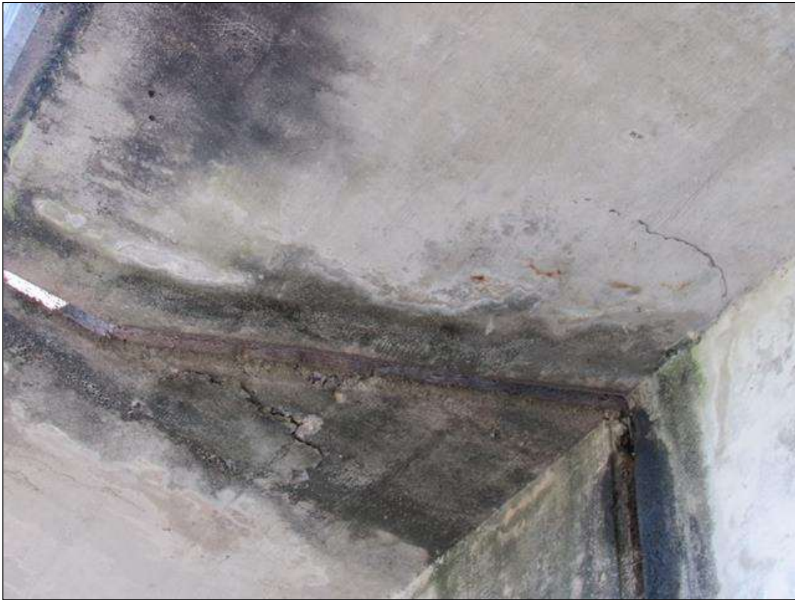
SPAN 3 FAR END & SPAN 4 NEAR END UNDESIDE OF DECK OVERHANG - DELAM (2SF), LEFT SIDE
