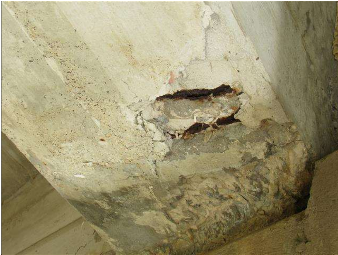
SPAN 4 BEAM 4 - SPALL (1FT X 8IN X 1.5IN) WITH EXPOSED REINFORCING TO BOTTOM AT FAR END
