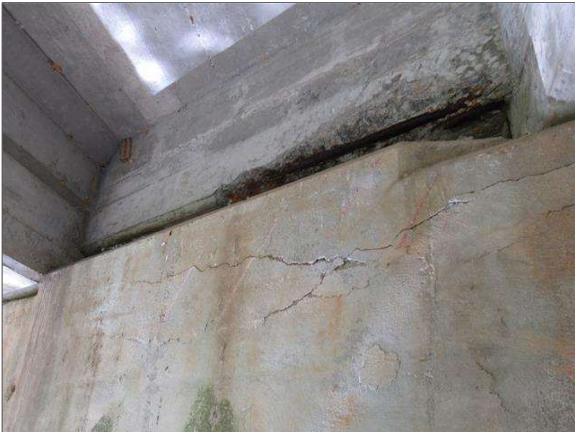
BENT 4 CAP, FAR FACE - DELAM (5SF) BAY 3 & SPALL (2.5FT X 8IN X 3IN) WITH EXPOSED REINFORCING TO SPAN 5 NEAR END DIAPHRAGM, BAY 3
