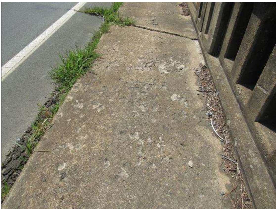
TYPICAL WEAR/SHALLOW SPALLING, (UP TO 1/2IN D.) WITH EXPOSED AGGREGATE THROUGHOUT SIDEWALK, SPAN 2 LEFT SIDE NEAR END
