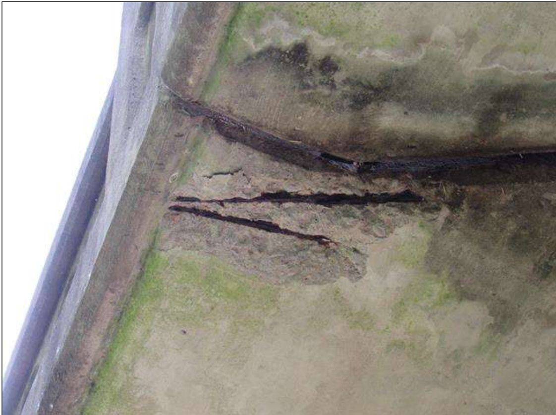
TYPICAL SPALL (UP TO 18IN X 12IN X 2IN) WITH EXPOSED REINFORCING TO UNDERSIDE OF DECK OVERHANG, SPAN 2 NEAR END
