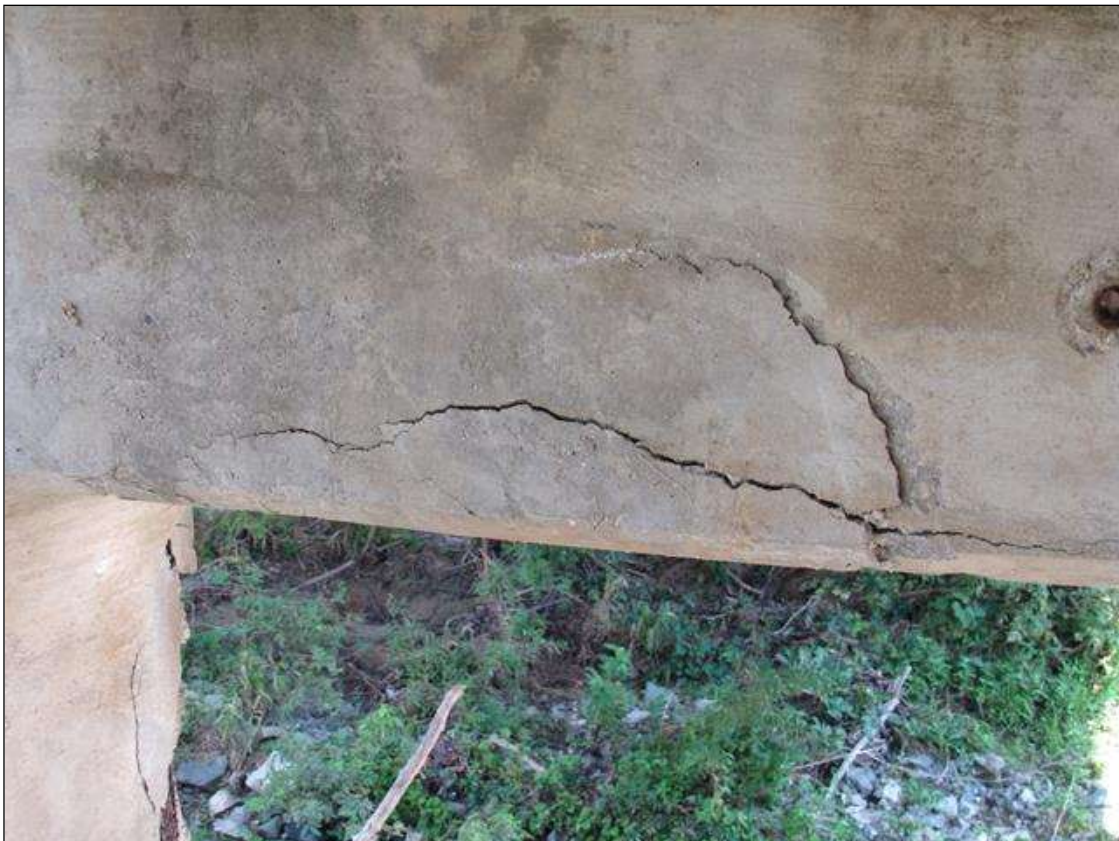
BENT 4 CAP, NEAR FACE - DELAM (3SF) TO GUSSET UNDER BEAM 1
