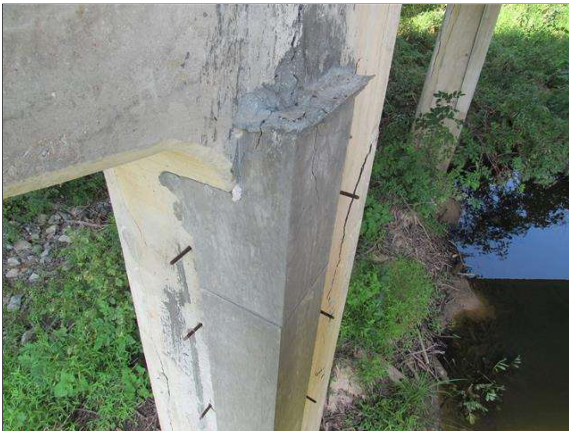
BENT 5 COLUMN 2 - DELAMINATED PATCH (10FT X 16IN) FAR RIGHT CORNER
