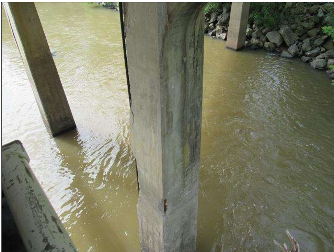
BENT 2 COLUMN 1 - DELAM/SPALL (8FT X 8IN X 3IN) WITH EXPOSED REINFORCING, STARTING 3FT FROM CAP, FAR LEFT CORNER
