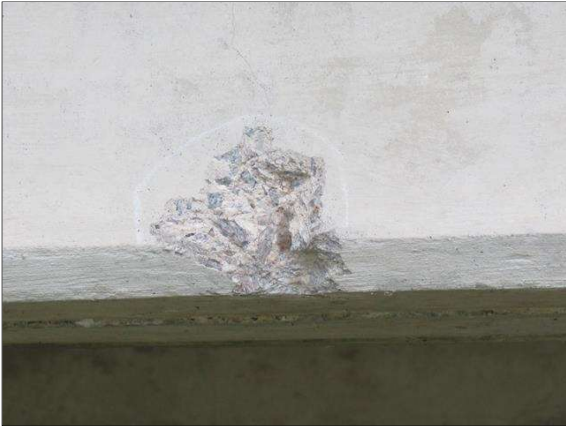
SPAN 1 BEAM 5 - SPALL (4IN X 4IN X 1IN) RIGHT SIDE AT BOTTOM, 15FT FROM NEAR END
