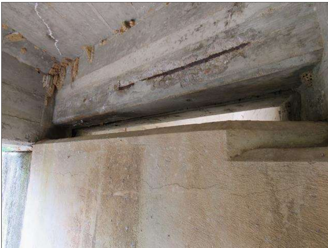
BENT 3 CAP FAR FACE - DELAM (5FT X 8IN) & SPALL (28IN X 6IN X 1IN) WITH EXPOSED REINFORCING, SPAN 4 NEAR END DIAPHRAGM, BAY 4
