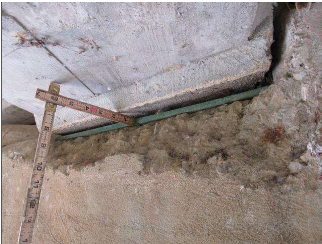
BENT 3 CAP, FAR FACE - SPALL (2FT X 6IN X 4IN) WITH BEARING LOSS, (UP TO 1.5IN X FULL W.) UNDER BEAM 2. REMAINING CONCRETE IS SOUND. (PAR PHOTO)
