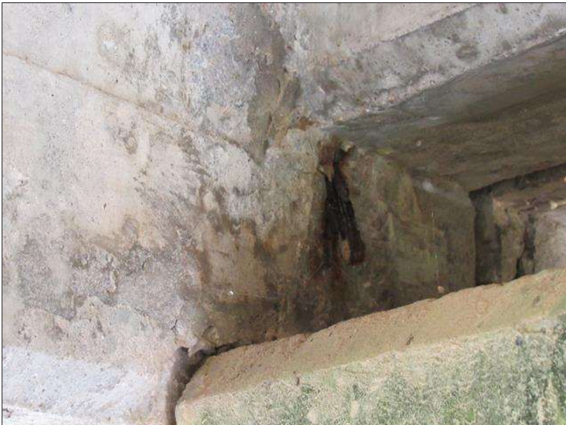
SPAN 3 BEAM 1 - SPALL (6IN X 1IN) WITH EXPOSED REINFORCING, RIGHT SIDE FAR END
