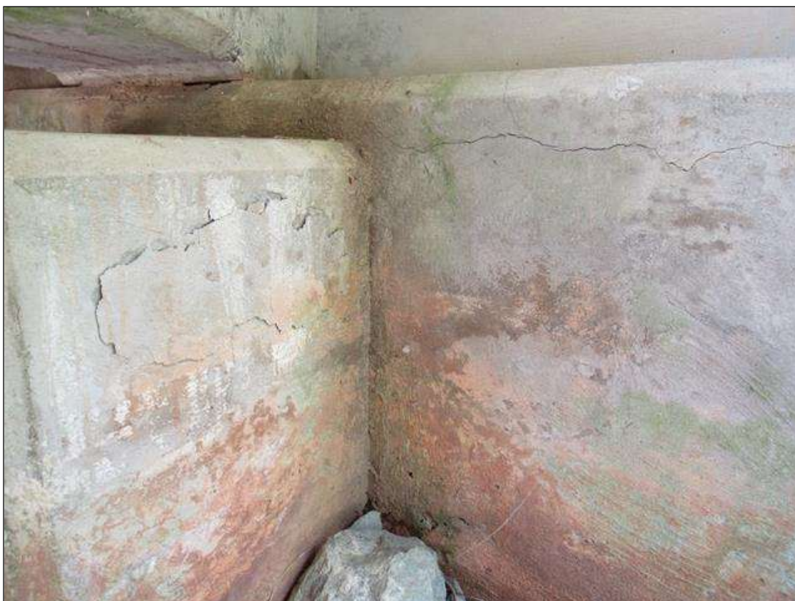
END BENT 2 CAP - DELAM (1FT X 6IN) TO LEFT END PILE CAP AT LEFT SIDE & LONGITUDINAL CRACK, (1/32IN X 2FT L.) LEFT OF BEAM 1
