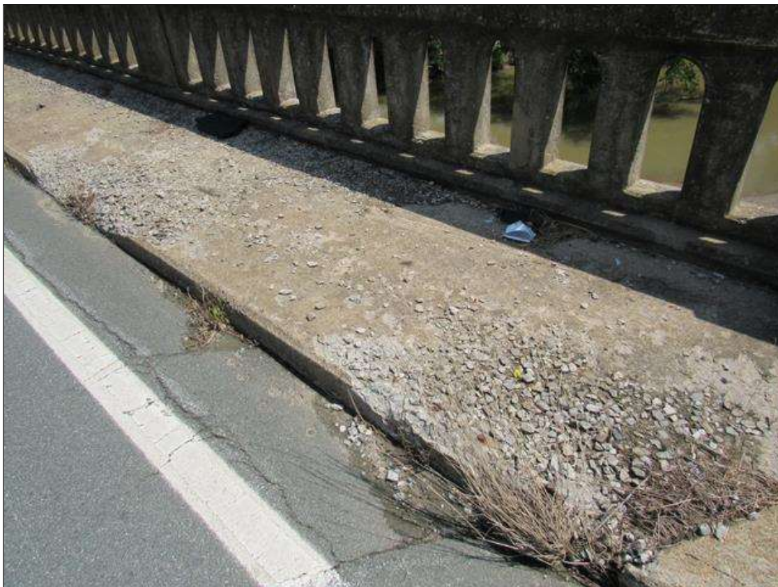
SPAN 3 SIDEWALK, RIGHT SIDE - SPALLING, (UP TO 5FT X 4FT X 4IN D.) WITH EXPOSED REINFORCING & LOOSE AGGREGATE, NEAR END. (PAR PHOTO)
