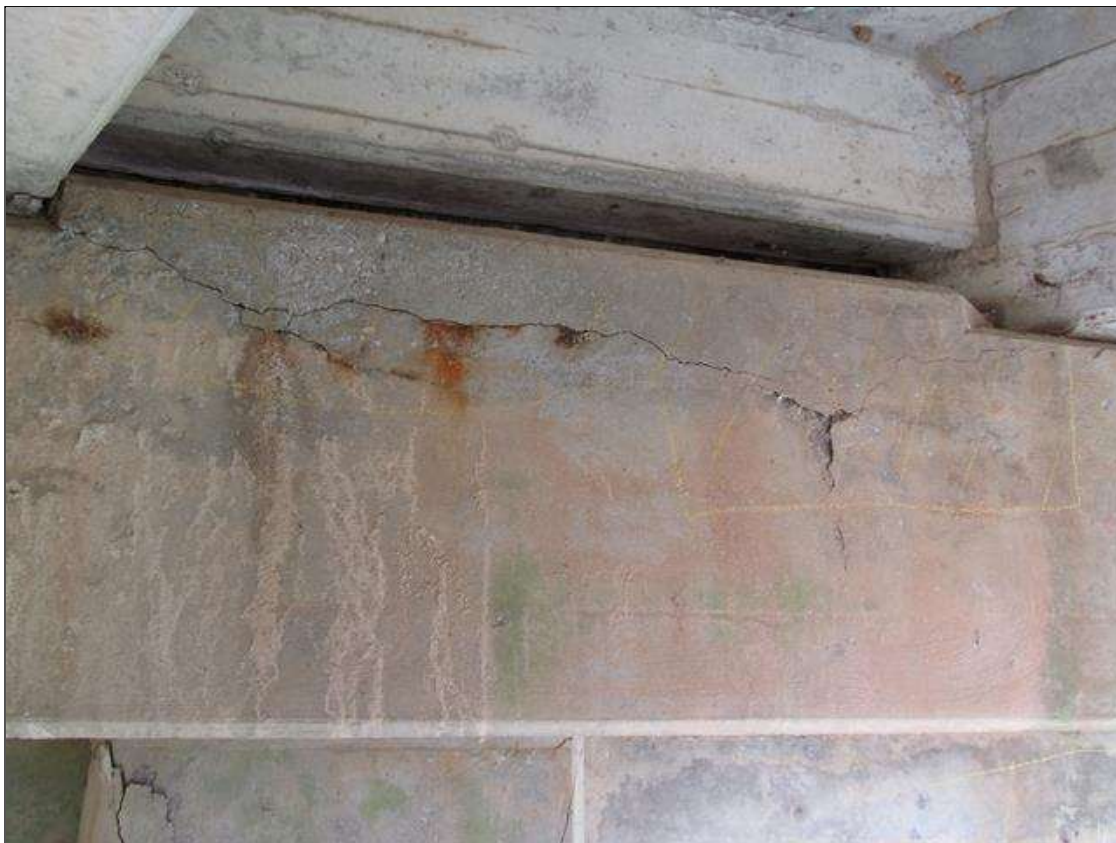
BENT 1 NEAR FACE - DELAM (5SF) ABOVE COLUMN 2
