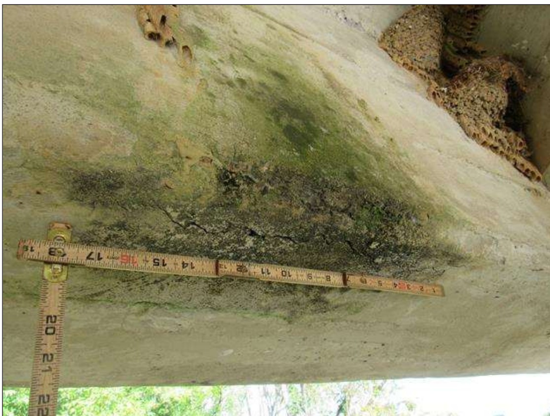
SPAN 2 BEAM 1 - DELAM (16IN X 8IN) BOTTOM RIGHT AT MID-SPAN
