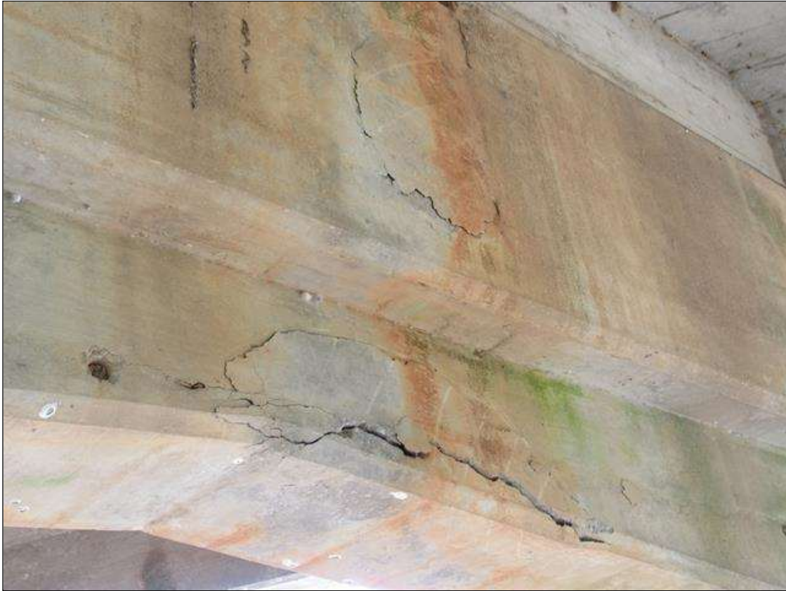
BENT 3, NEAR FACE - (X2) DELAM (UP TO 3SF) UNDER BEAM 3
