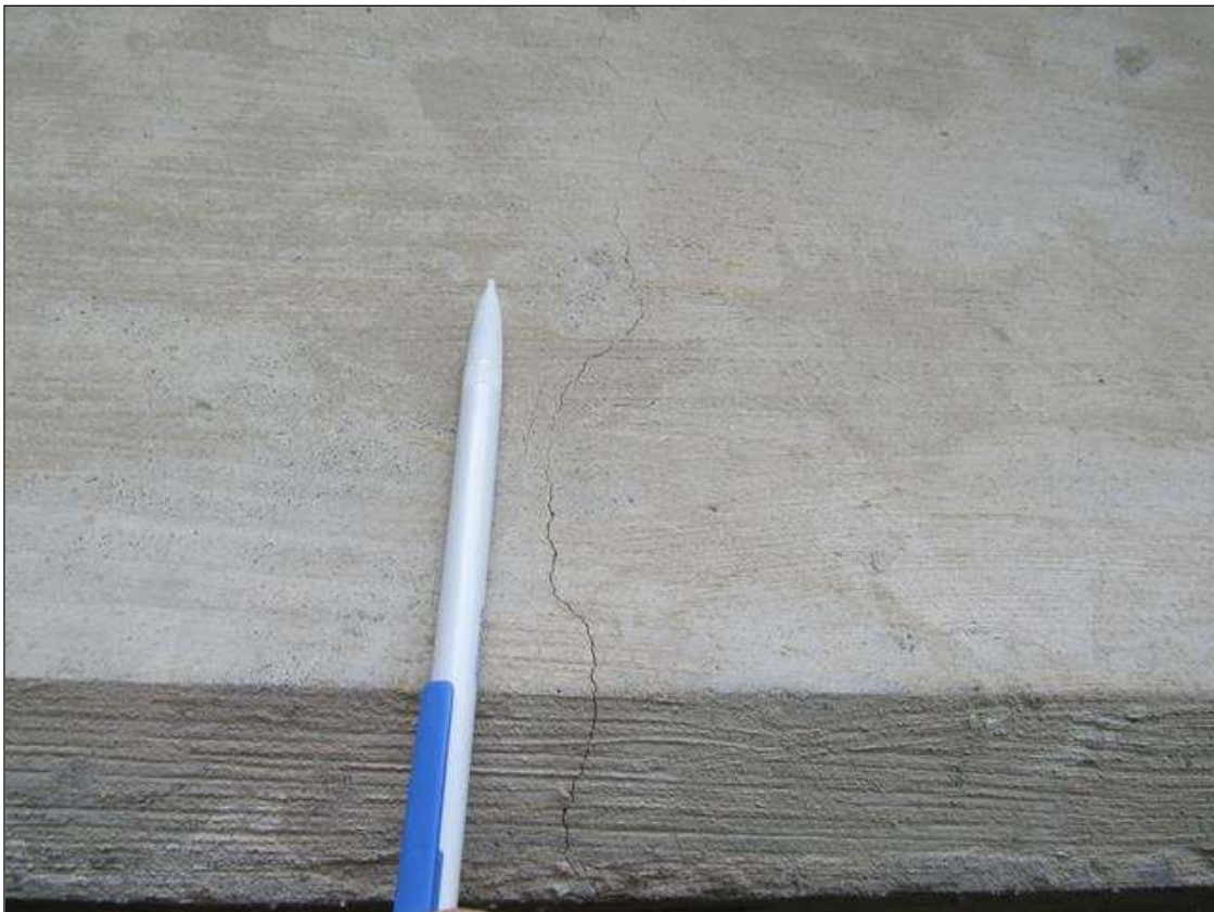
TYPICAL INTERMITTENT VERTICAL HAIRLINE CRACKING, (UP TO FULL HT.) SPACED UP TO 2FT O.C. THROUGHOUT BEAMS, SPAN 1 BEAM 5 MID-SPAN
