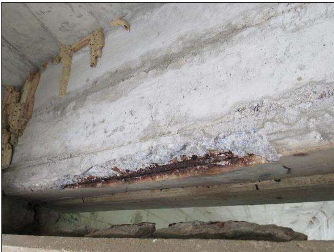
SPAN 2 NEAR END DIAPHRAGM, BAY 2 - SPALL (28IN X 4IN X 2IN) WITH EXPOSED REINFORCING
