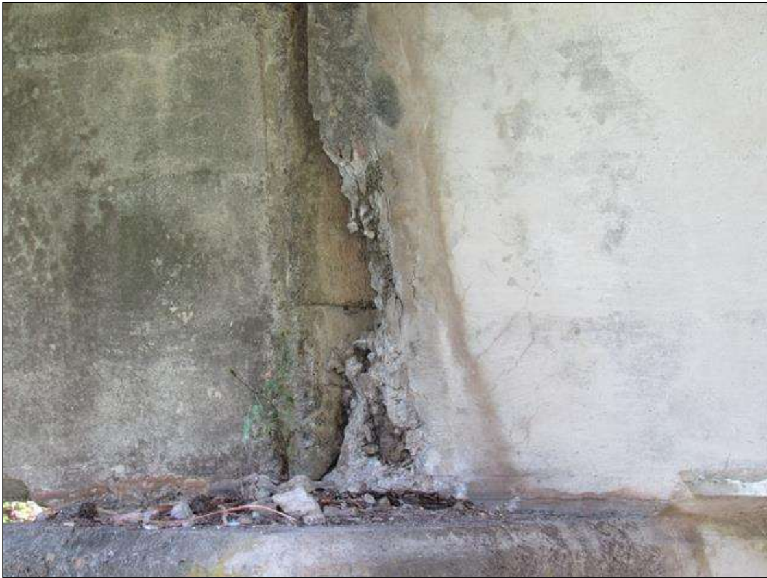
SPAN 5 BEAM 1 - SPALL (18IN X 6IN X 3IN) NO EXPOSED REINFORCING, FAR END LEFT SIDE
