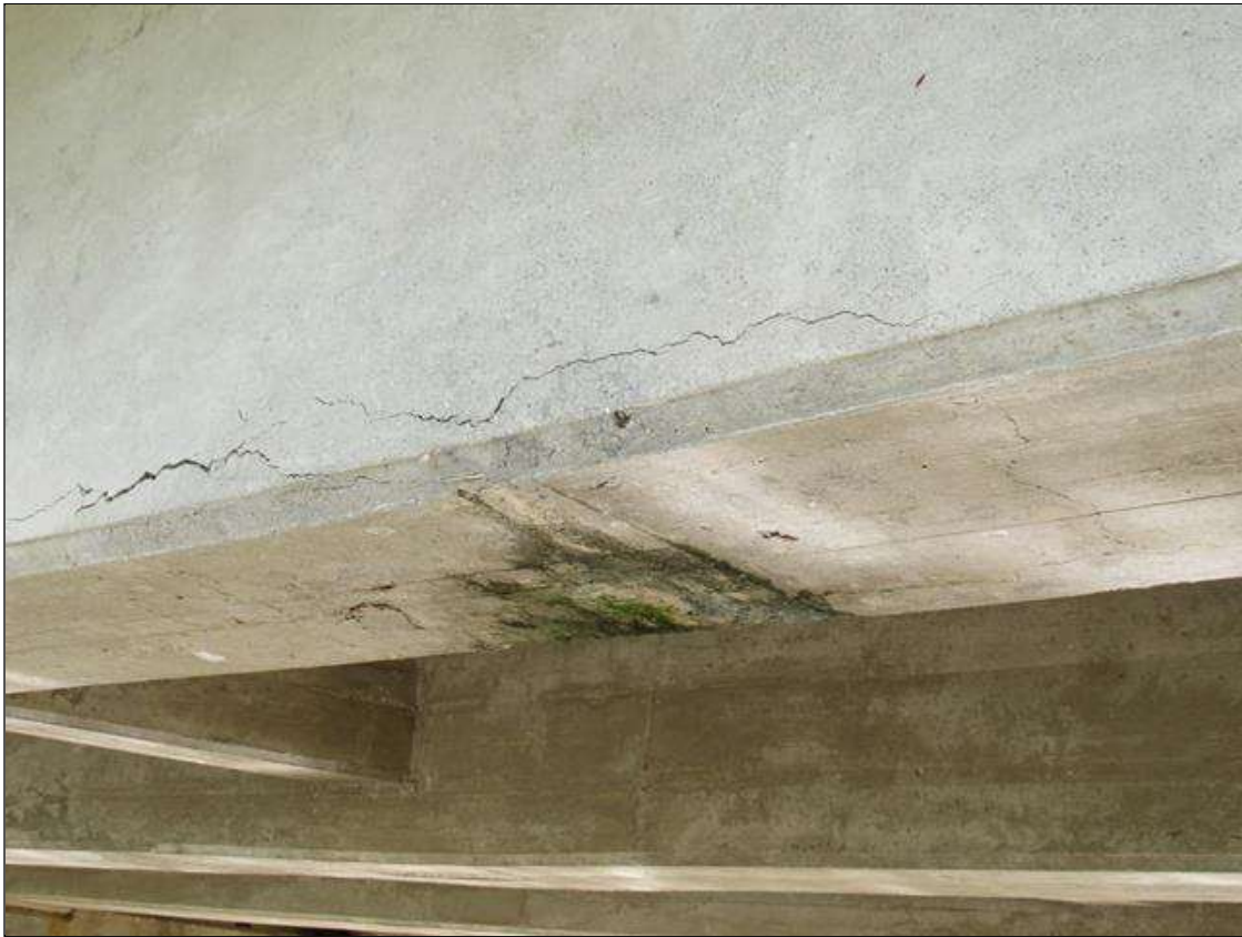
SPAN 4 BEAM 1 - DELAM (4FT X FULL W.) BOTTOM OF BEAM 12FT FROM NEAR END
