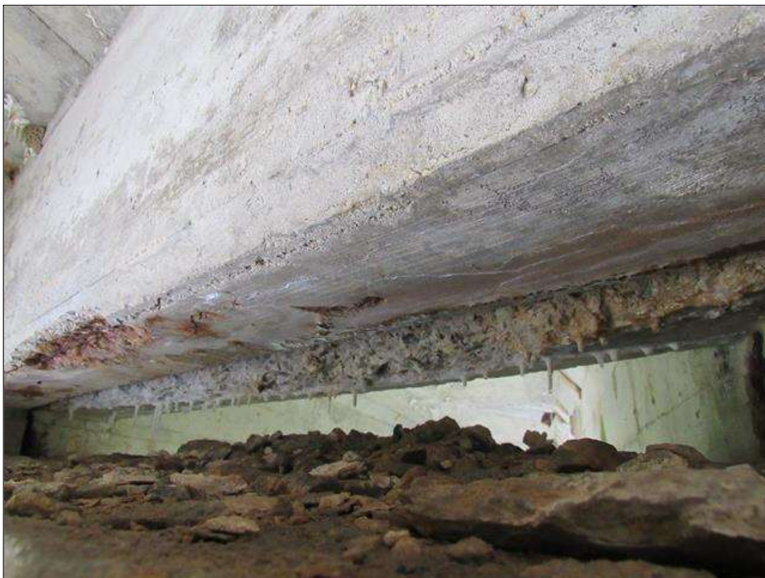
SPAN 1 FAR END, SPAN 2 NEAR END DIAPHRAGM, BAY 1 - SPALL (5FT X 6IN X 3IN) WITH EXPOSED REINFORCING & HEAVY EFFLO.
