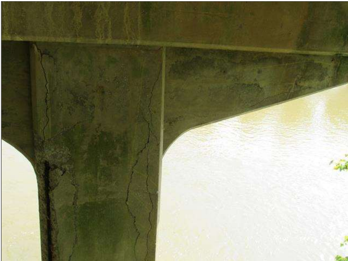
BENT 1 CAP & COLUMN , NEAR FACE - DELAM (6FT X 1FT) NEAR RIGHT CORNER & (3SF) AT RIGHT GUSSET
