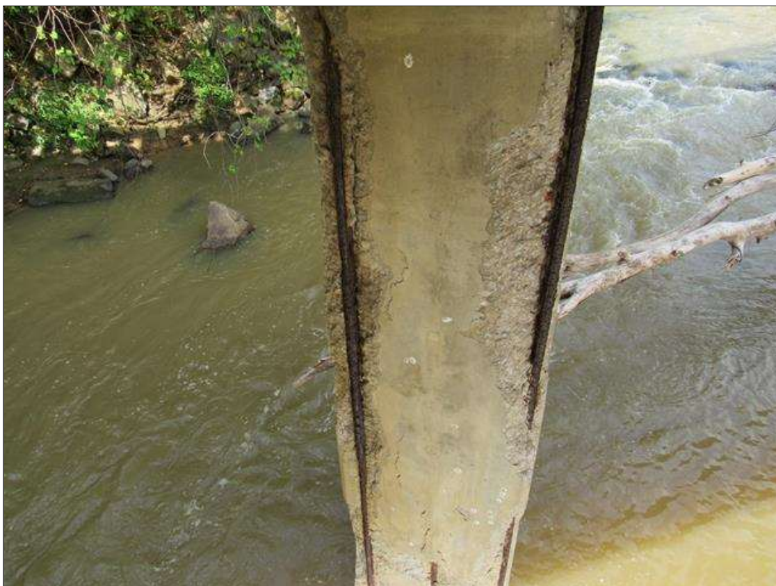
BENT 2 COLUMN 1, RIGHT SIDE - SPALL/DELAM (UP TO 25FT L. X 3FT W. X 6IN D.) WITH EXPOSED REINFORCING. (PAR PHOTO)
