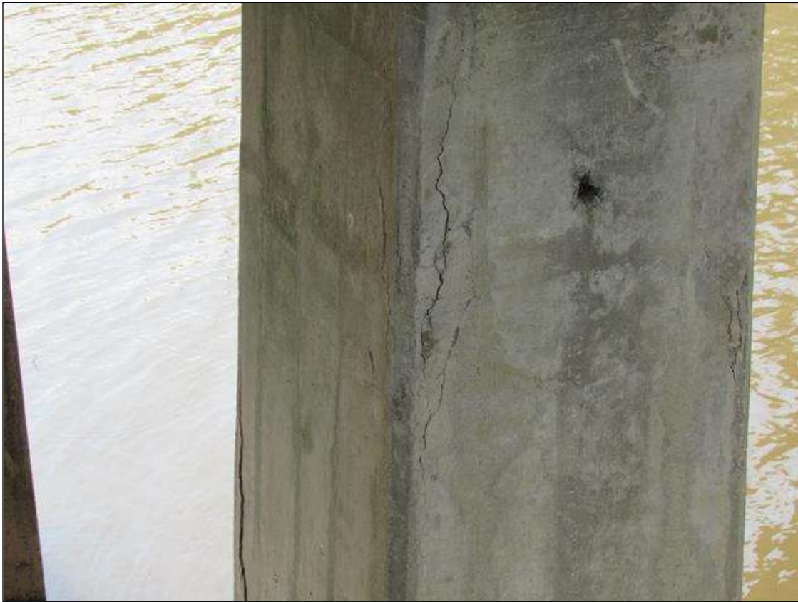
BENT 3 COLUMN 1 - DELAM (3FT X 6IN) FAR LEFT CORNER STARTING 4FT FROM CAP
