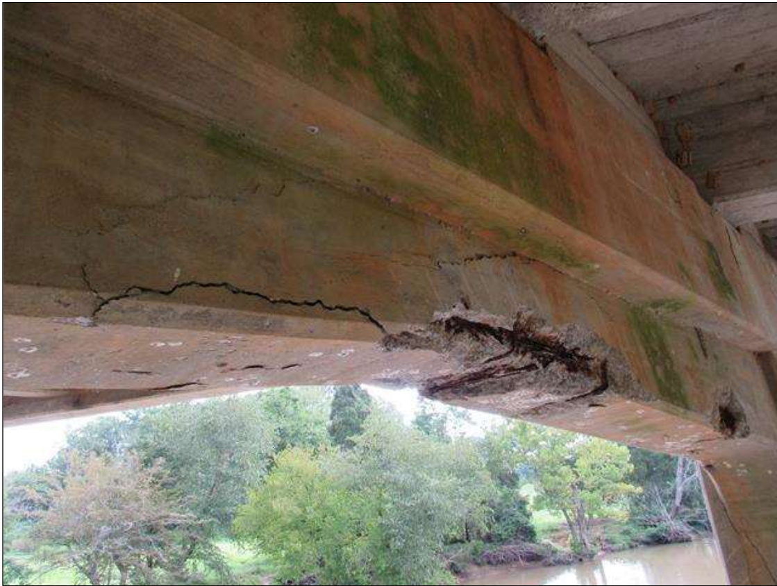
BENT 2 CAP, NEAR FACE - SPALL/DELAM (UP TO 7FT X 2FT X 5IN) WITH EXPOSED REINFORCING. (PAR PHOTO)
