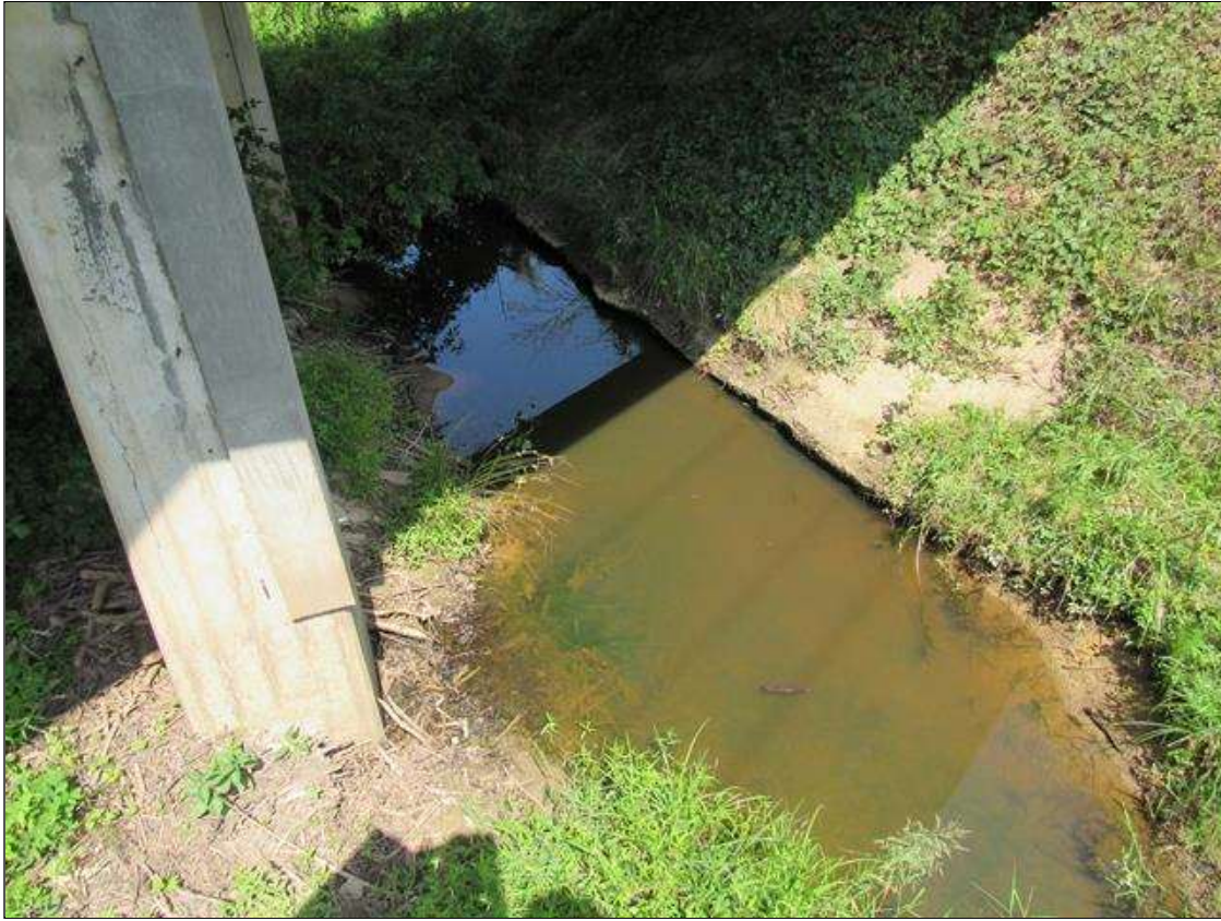
EROSION HOLE (50FT L. X 12FT W. X 2FT D.) AT BASE OF END BENT 2 SLOPE PROTECTION
