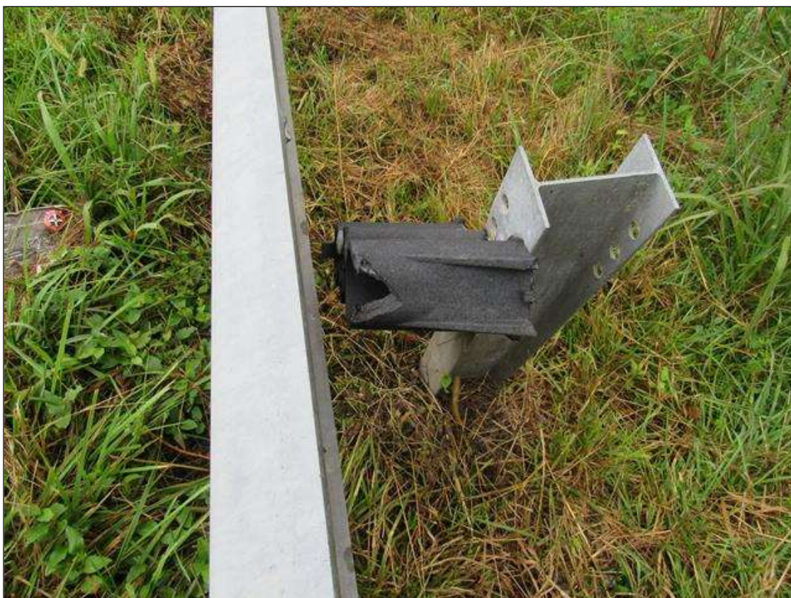
NEAR RIGHT GUARDRAIL POST - POST NOT ATTACHED, POST 8 FROM END TREATMENT, POST 3 & 5 SIMILAR
