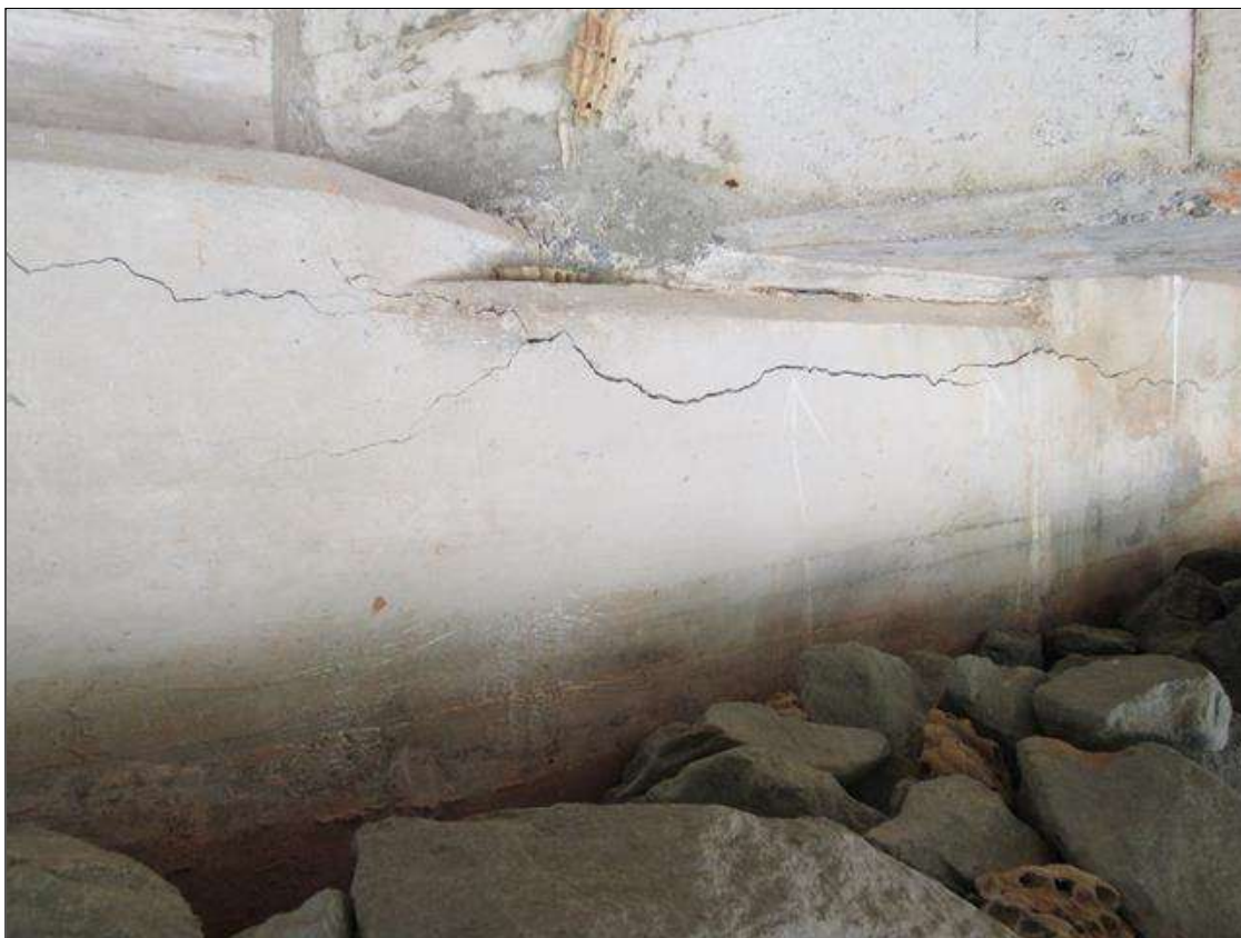
END BENT 1 CAP - LONGITUDINAL OPEN CRACK, (1/8IN X 5FT L.) UNDER BEAM 2
