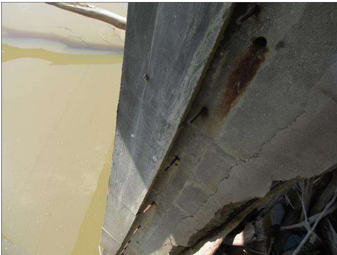
BENT 4 COLUMN 2 - PARTIALLY DELAMINATED PATCH, (2SF) AT TOP, FAR RIGHT CORNER
