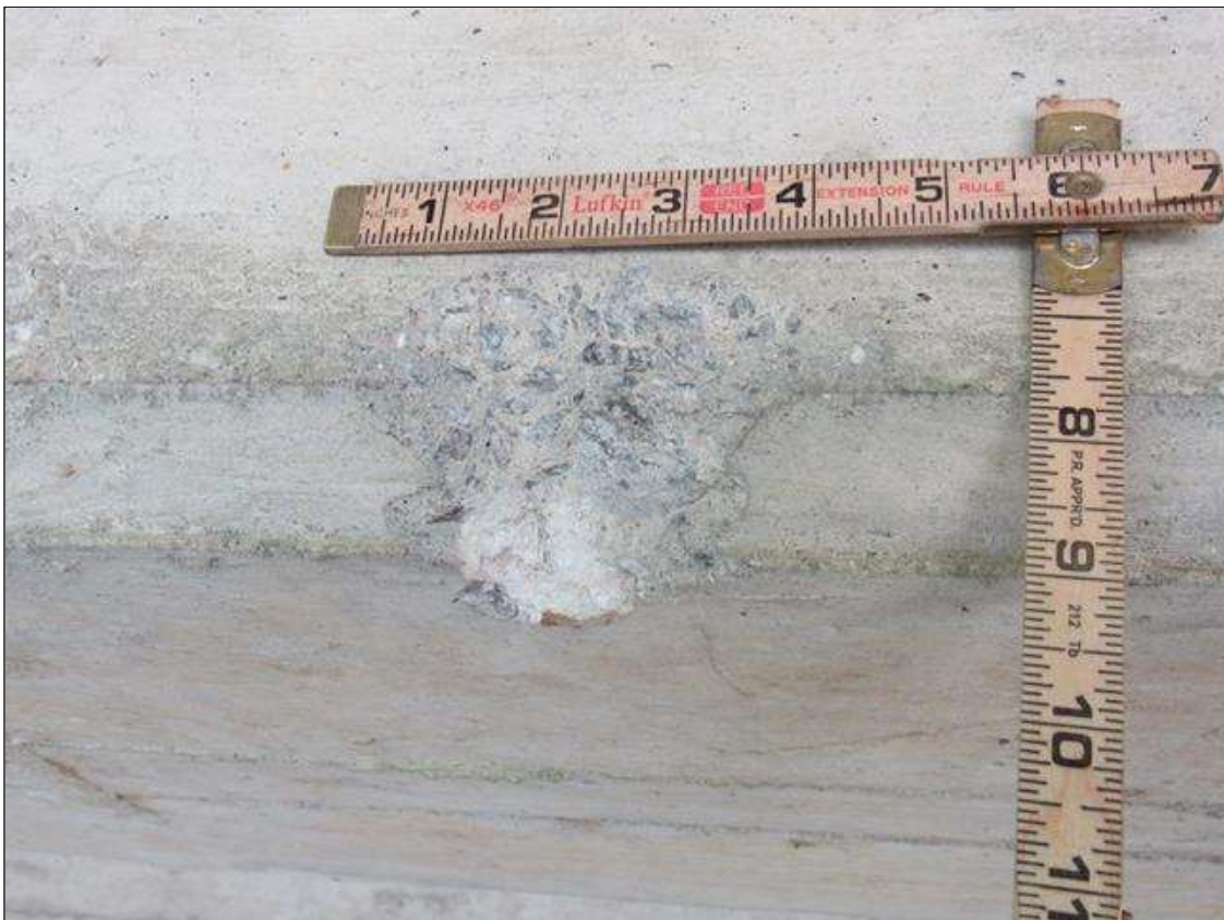
SPAN 1 BEAM 3 - SPALL ( 3IN X 3IN X 1/2IN) BOTTOM RIGHT, MID-SPAN
