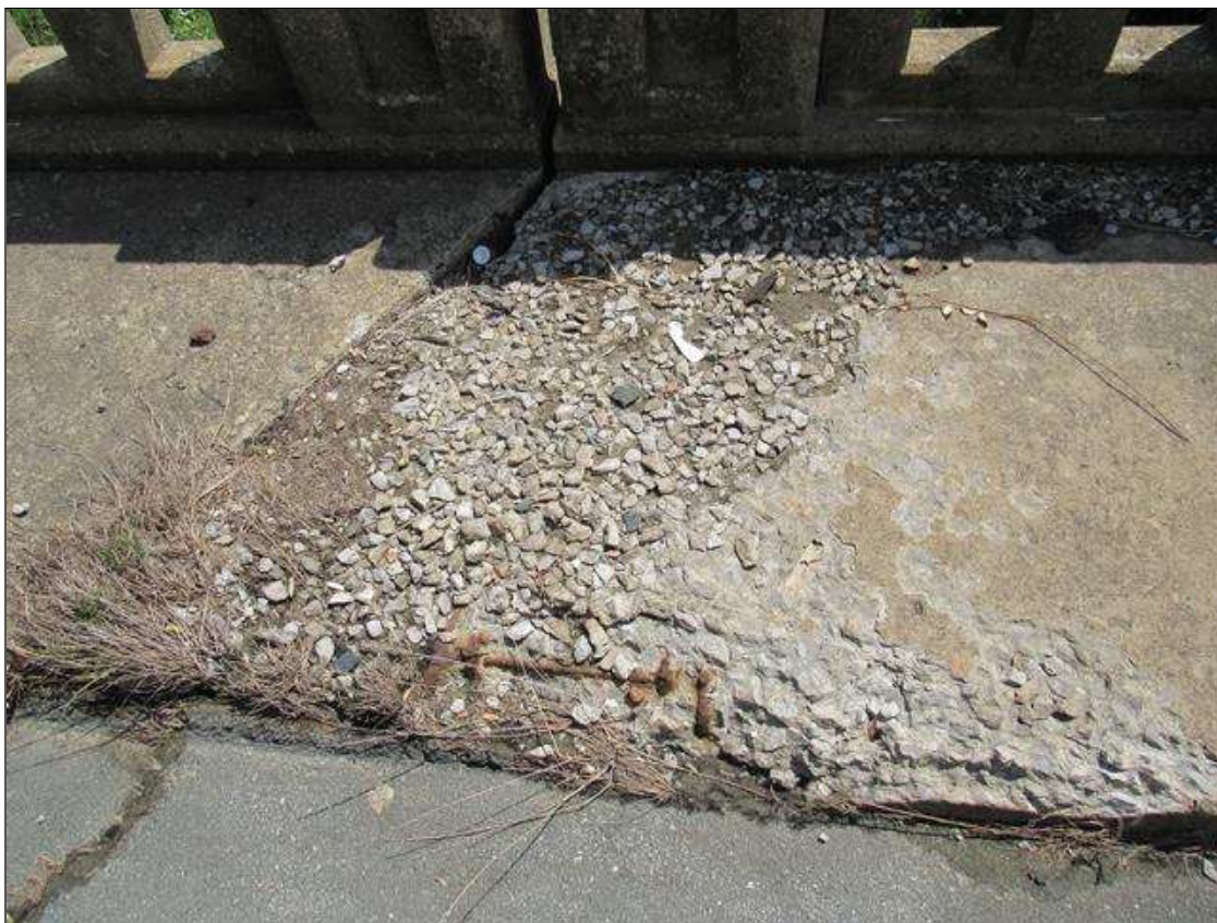
SPAN 5 SIDEWALK, RIGHT SIDE - SPALLING, (UP TO 4FT X 4FT X 4IN) WITH EXPOSED REINFORCING & LOOSE AGGREGATE, FAR END. (PAR PHOTO)
