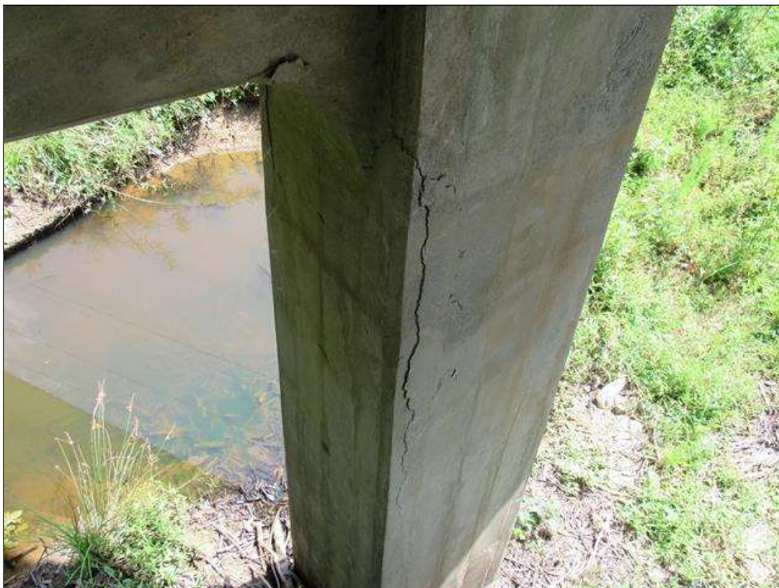
BENT 5 COLUMN 2 - DELAM (10FT X 1FT) NEAR LEFT CORNER STARTING AT TOP OF COLUMN
