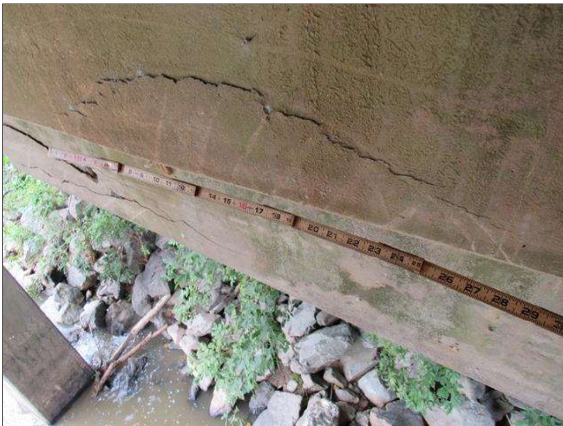
BENT 1 CAP, FAR FACE - DELAM (30IN X 7IN) BOTTOM EDGE UNDER BAY 2
