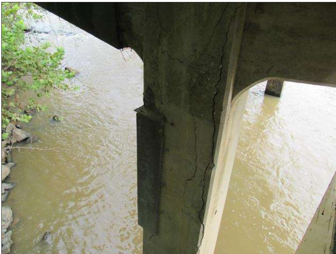
BENT 1 COLUMN 1 - DELAM (12SF) NEAR RIGHT CORNER, STARTING AT TOP OF COLUMN
