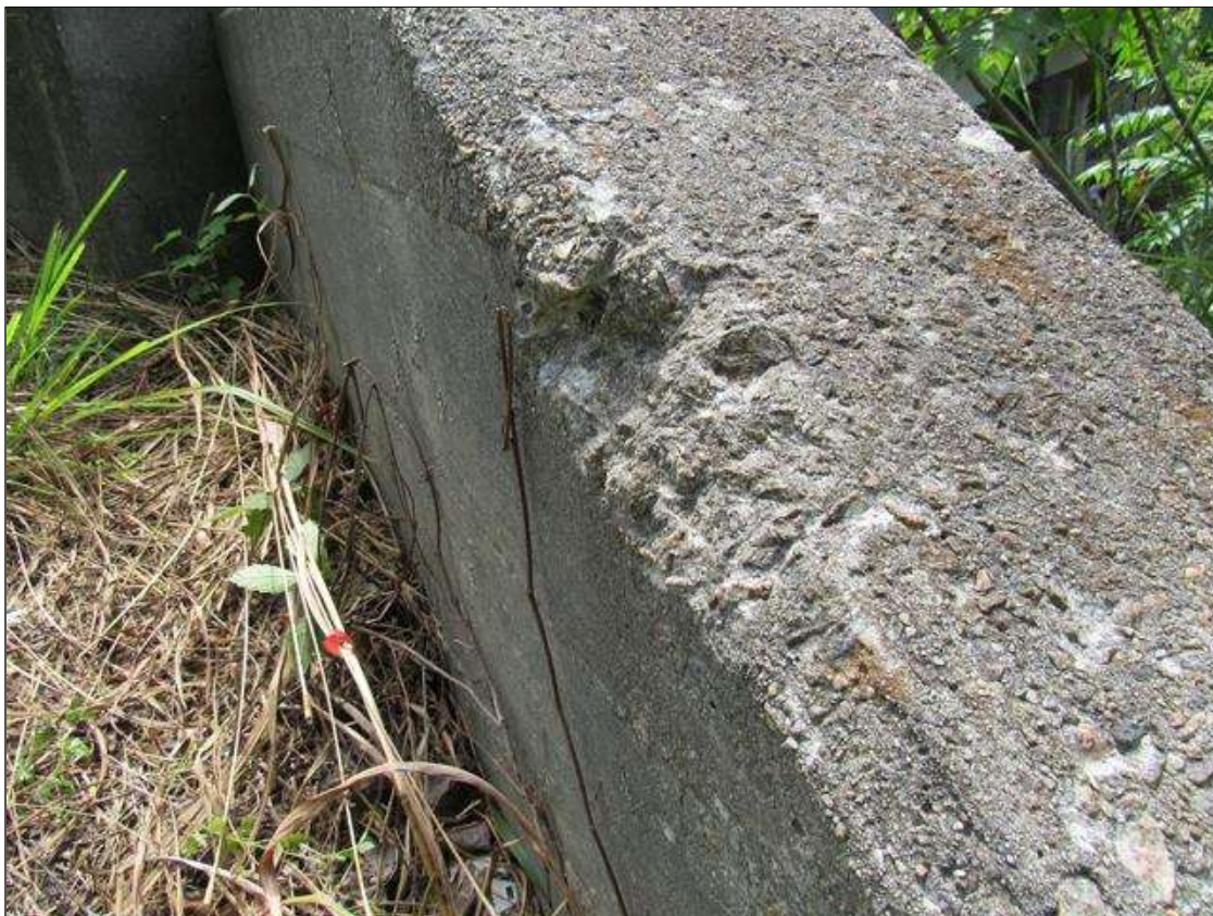
FAR LEFT WINGWALL - SPALL (7IN X 4IN X 3/4IN) NO EXPOSED REINFORCING, FAR CORNER
