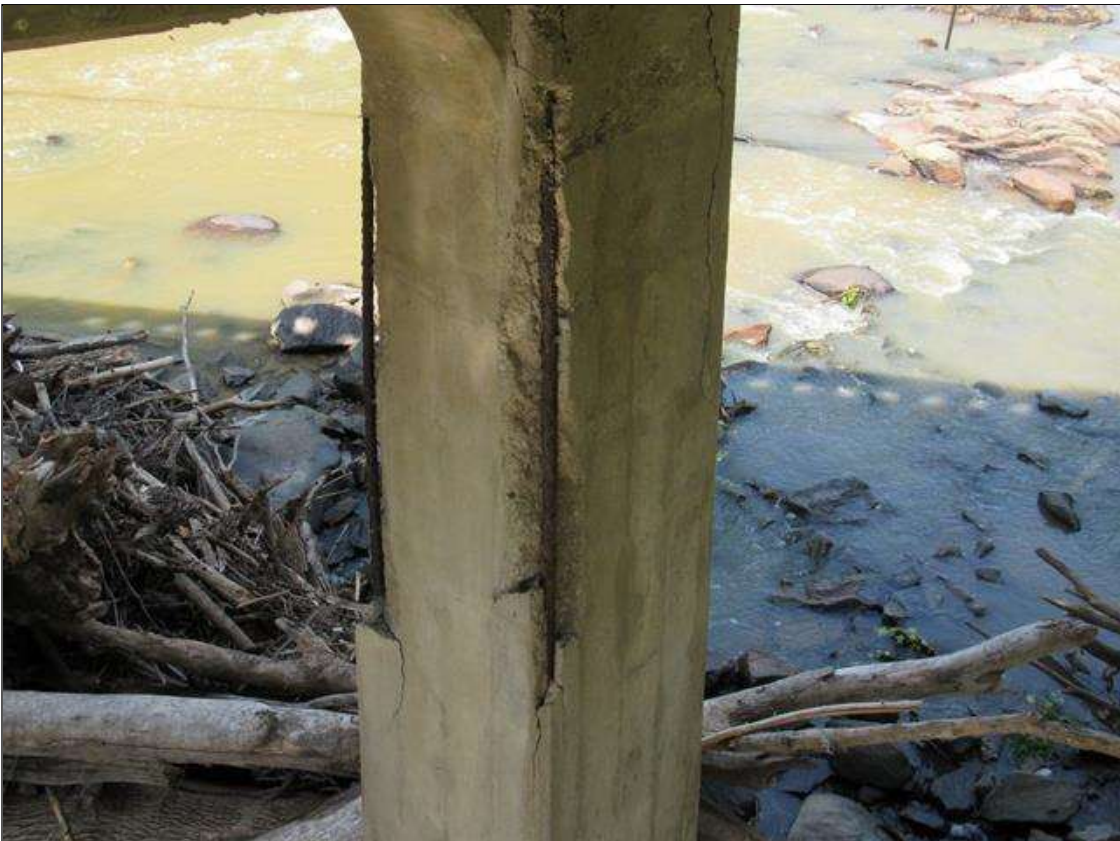
BENT 4 COLUMN 1 - SPALLING/DELAM (10FT L. X 1FT W. X 4IN D.) WITH EXPOSED REINFORCING, FAR & NEAR RIGHT CORNER. (PAR PHOTO)
