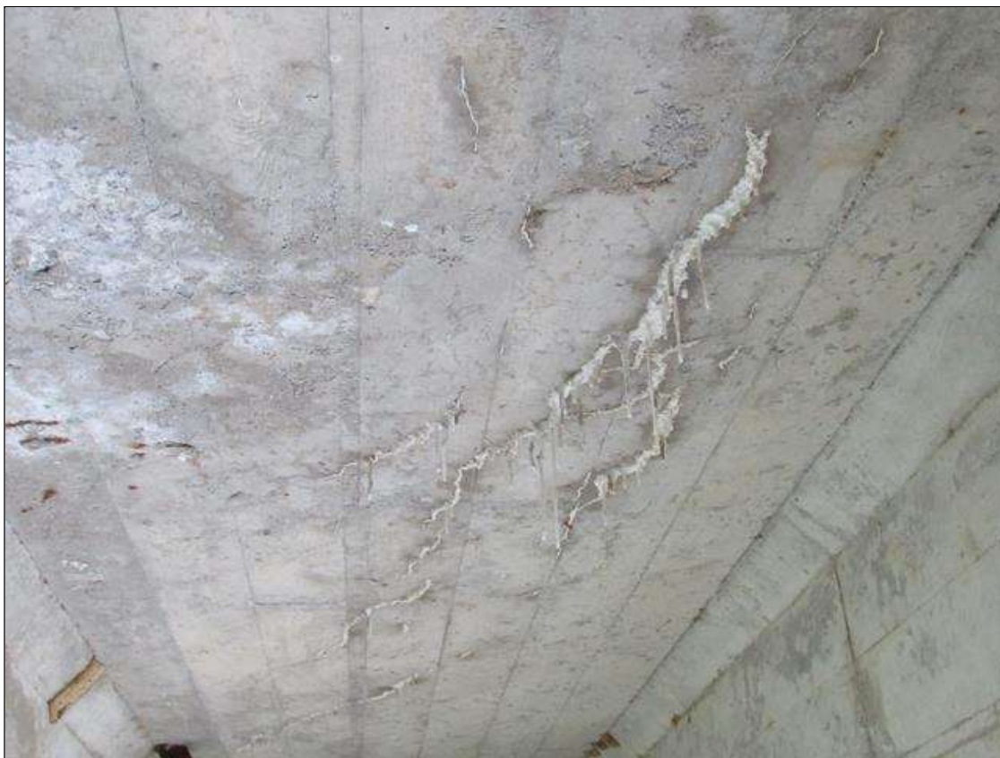
TYPICAL INTERMITTENT HAIRLINE TO 1/32IN LONGITUDINAL CRACKING WITH MODERATE TO HEAVY EFFLO. THROUGHOUT UNDERSIDE OF DECK, SPAN 1 BAY 1
