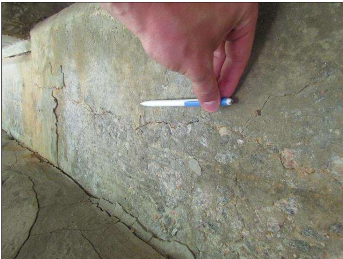
TYPICAL INTERMITTENT LONGITUDINAL HAIRLINE TO 1/32IN CRACK, (UP TO 5FT L.) THROUGHOUT CAP, END BENT 2 BAY 4
