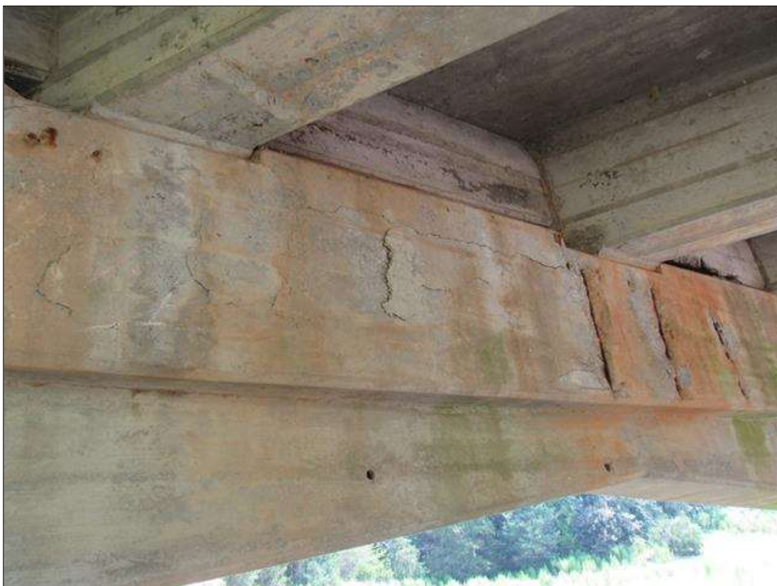
BENT 5 CAP, NEAR FACE - INTERMITTENT DELAM/SPALLING, (UP TO 3SF X 2IN D.) WITH EXPOSED REINFORCING, BETWEEN BEAMS 2 & 3
