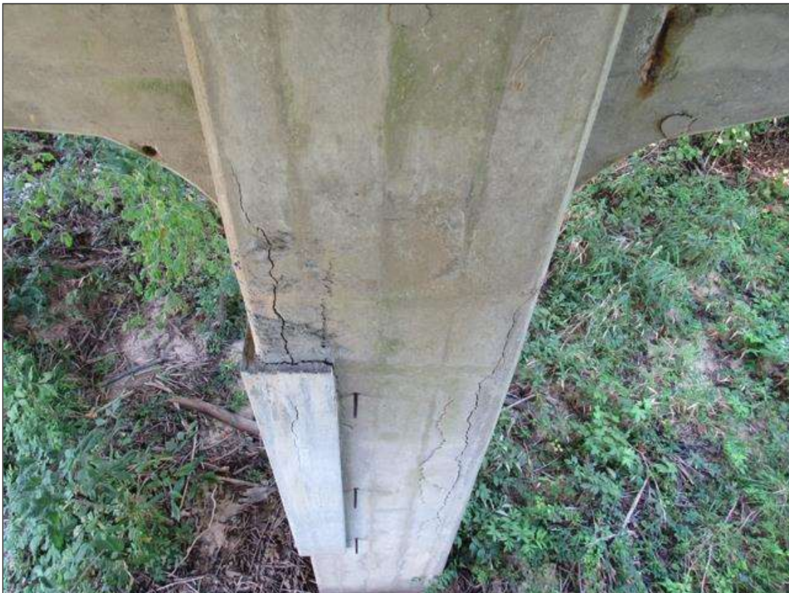
BENT 5 COLUMN 1 - DELAMINATED PATCH (8FT X 16IN) FAR RIGHT CORNER & DELAM (10FT X 1FT) FAR LEFT CORNER
