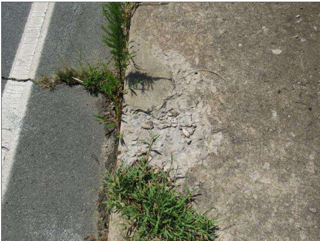
SPAN 5 SIDEWALK, LEFT SIDE - SPALLING, (3FT X 2FT X 1.5IN) WITH EXPOSED REINFORCING & LOOSE AGGREGATE, FAR END
