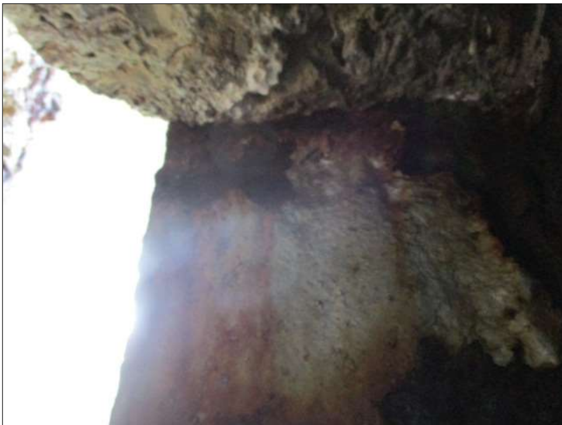
Span 2 Beam 9: PAR: 3/8" REMAINING (1/4" SECTION LOSS) ON TOP 2 1/2" OF WEB FOR 8" LONG UNDER DIAPHRAGM AT BENT 2
