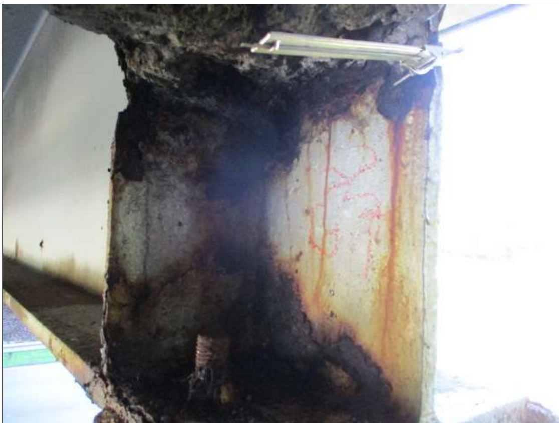
Span 2 Beam 1: PAR: 3/8" REMAINING (1/4" SECTION LOSS) ON TOP 3" OF WEB FOR 8" LONG UNDER DIAPHRAGM AT BENT 2
