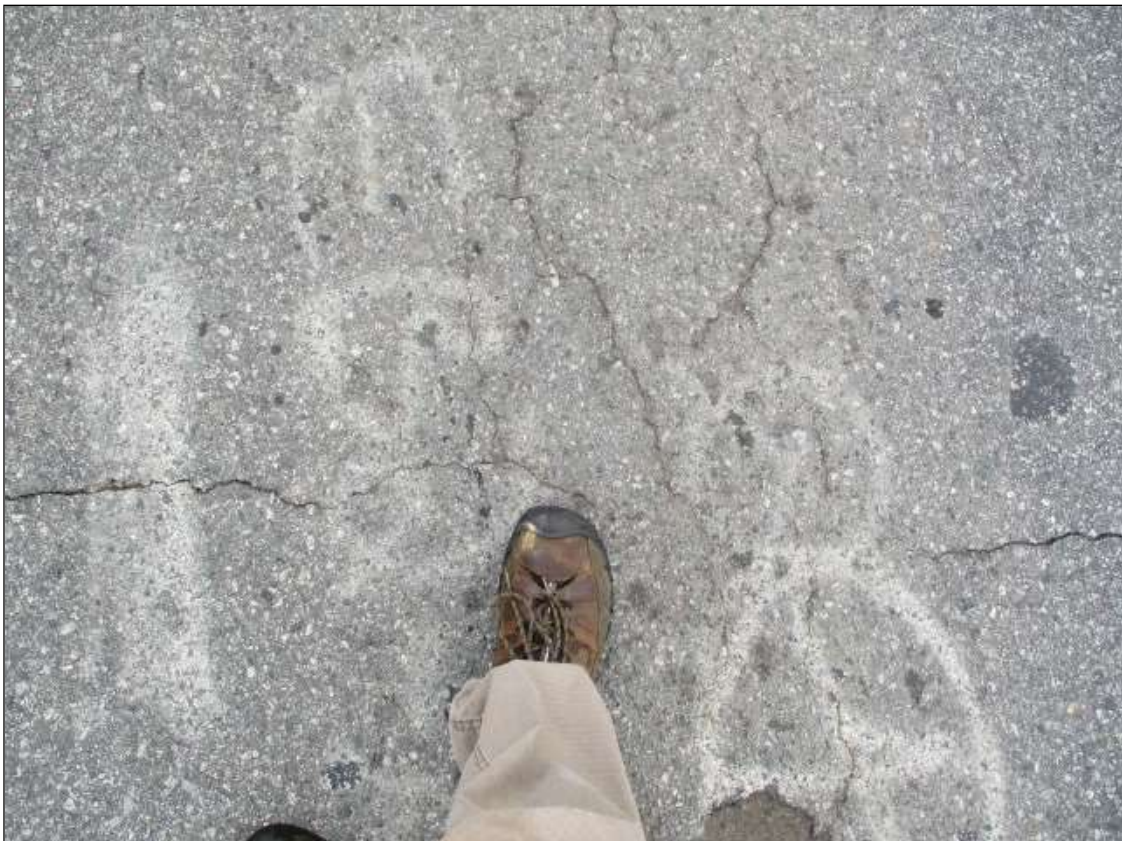
Span 3 Wearing Surface: 1/8" wide map cracking thru out the top of the wearing surface
