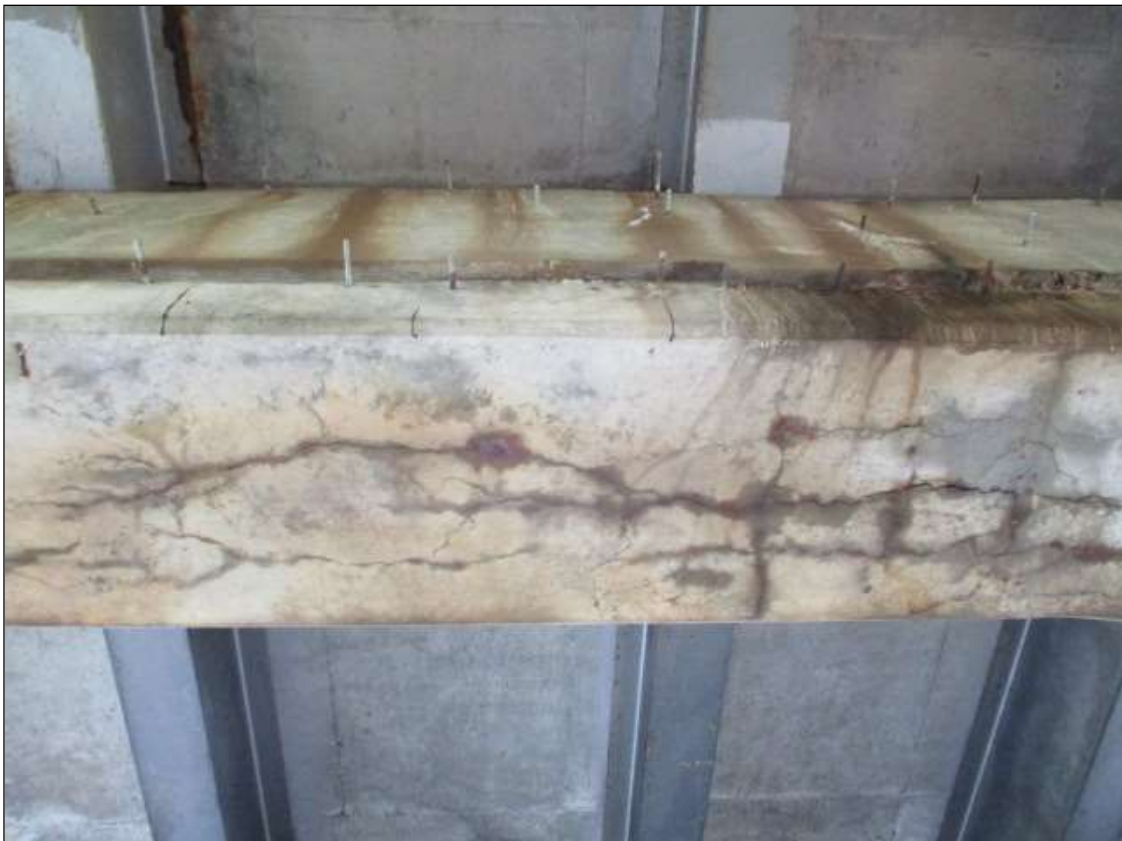
Bent 1 Cap 1: 1/32" MAP CRACKING THROUGHOUT UNDERSIDE
