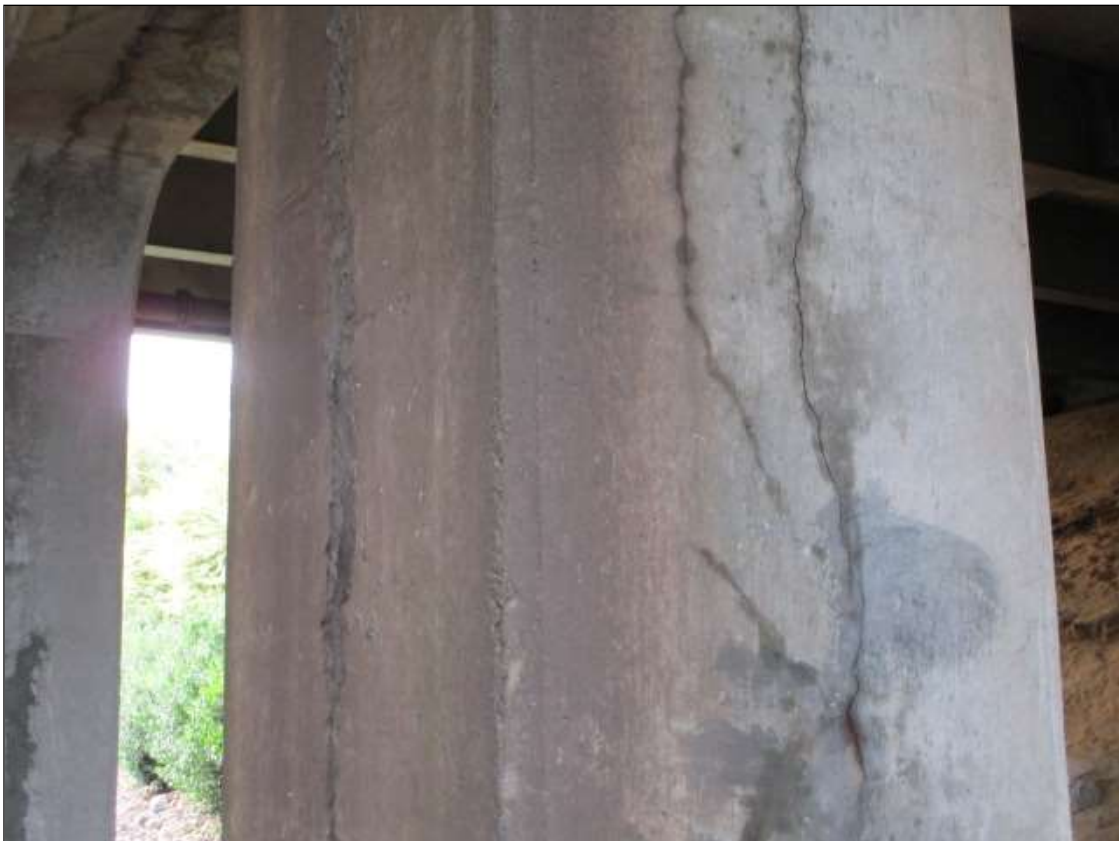
Bent 1 Pile 2: 1/16" wide cracking and unsound patches on all sides, full height
