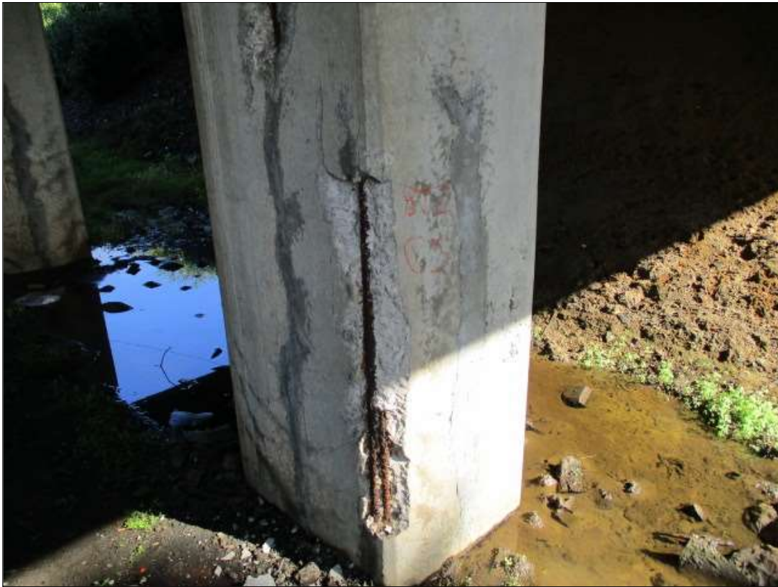
Bent 2 Pile 3: PAR: 4' X 8" X 6" SPALL WITH EXPOSED REBAR WITH SECTION LOSS ON SOUTHWEST CORNER
