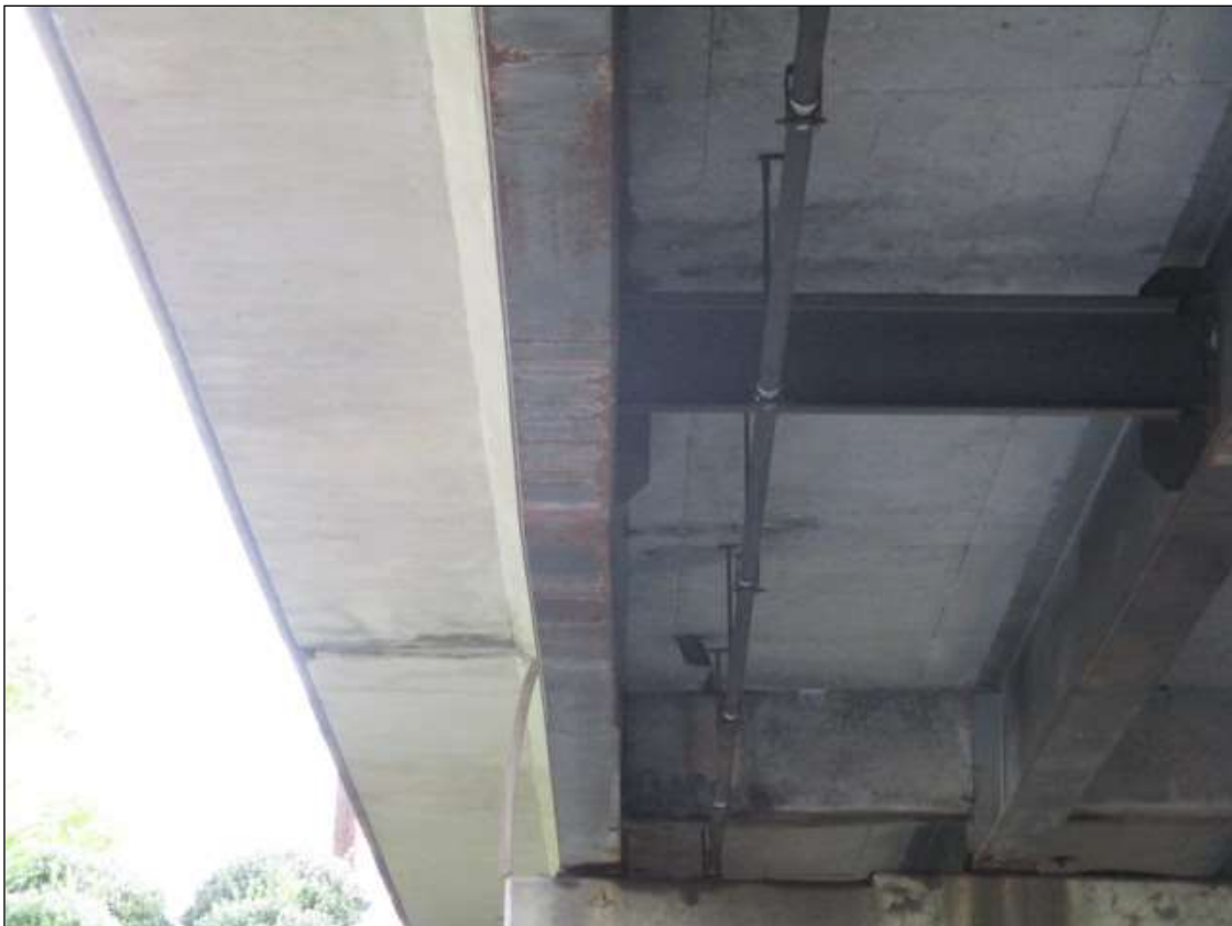
Span 2 Beam 1: at 22ft-9in from Bent 2, impact damage - lower web pushed out 1in x 8in high with divot on bottom flange [3/16in deep] and bottom flange bent upwards [1/4in]
