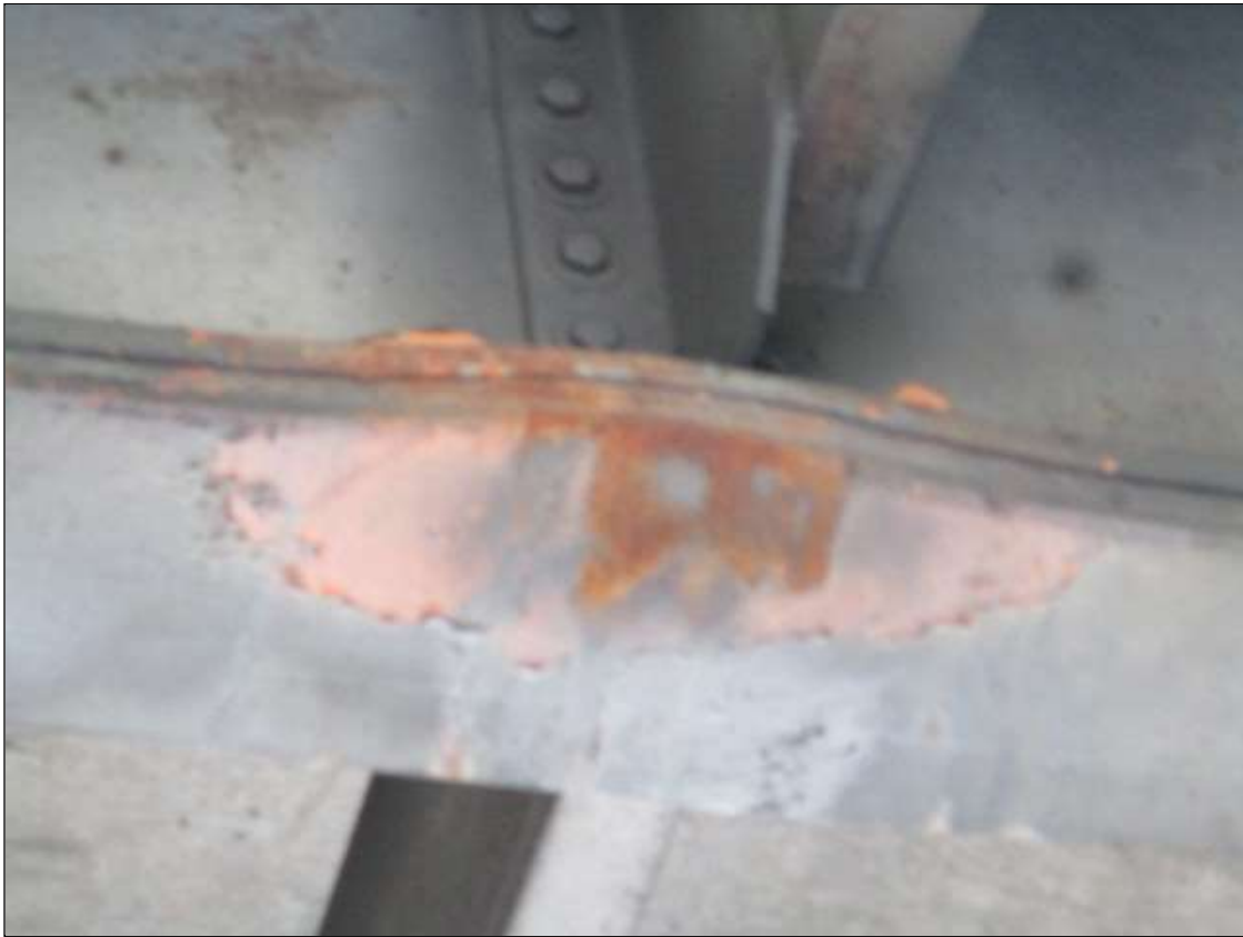
Span 2 Beam 4: PAR: at 22ft-11in from bent 1 bearing, impact damage - bottom flange bent upward 2-1/2in with lower web buckled [up to 1-1/2in] and gouge in cover plate [1/8in deep]
