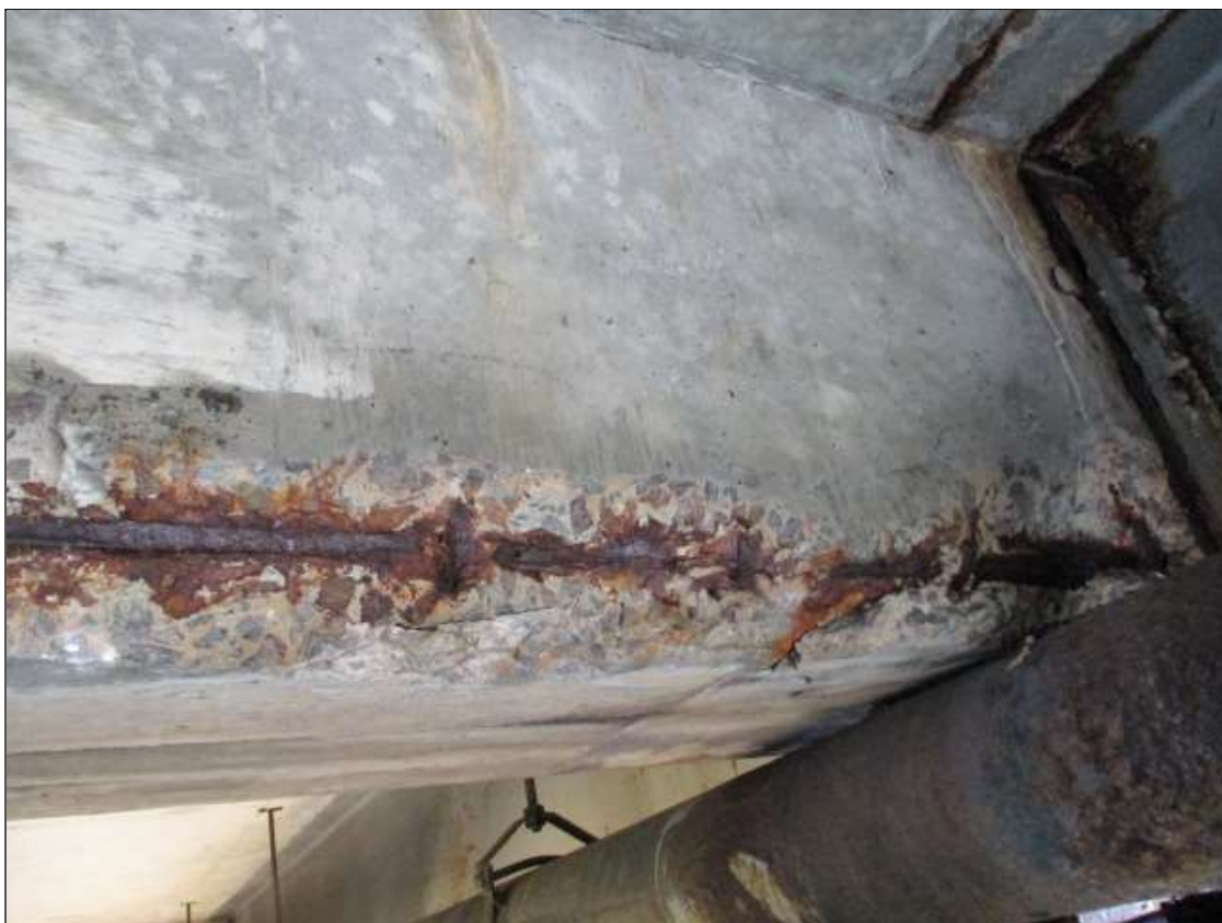
Span 2 Deck: PAR: 5' X 8" X 5" SPALL WITH EXPOSED REBAR WITH SECTION LOSS IN BAY 8 DIAPHRAGM OVER BENT 2
