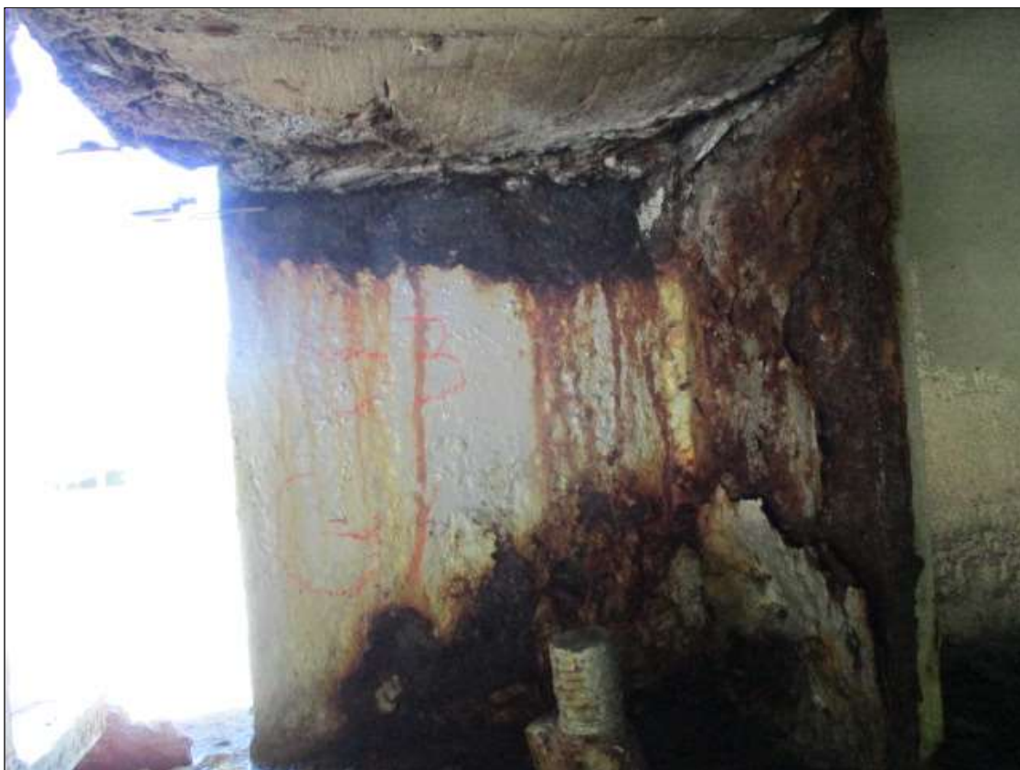
Span 3 Beam 1: PAR: 7/16" REMAINING (3/16" SECTION LOSS) ON TOP 2" OF WEB FOR 8" LONG UNDER DIAPHRAGM AT BENT 2
