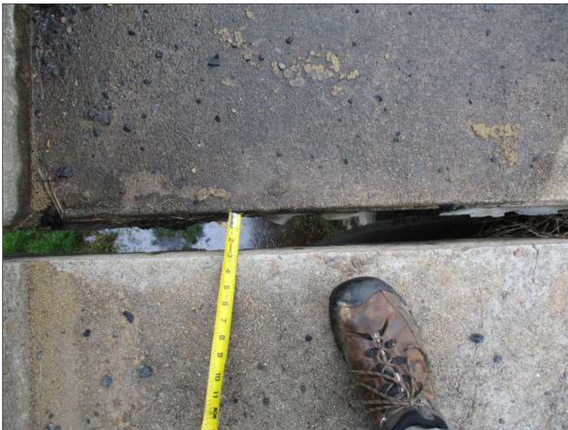
MISSING JOINT MATERIAL IN SIDEWALKS OVER INTERIOR BENTS WITH 3" GAP
