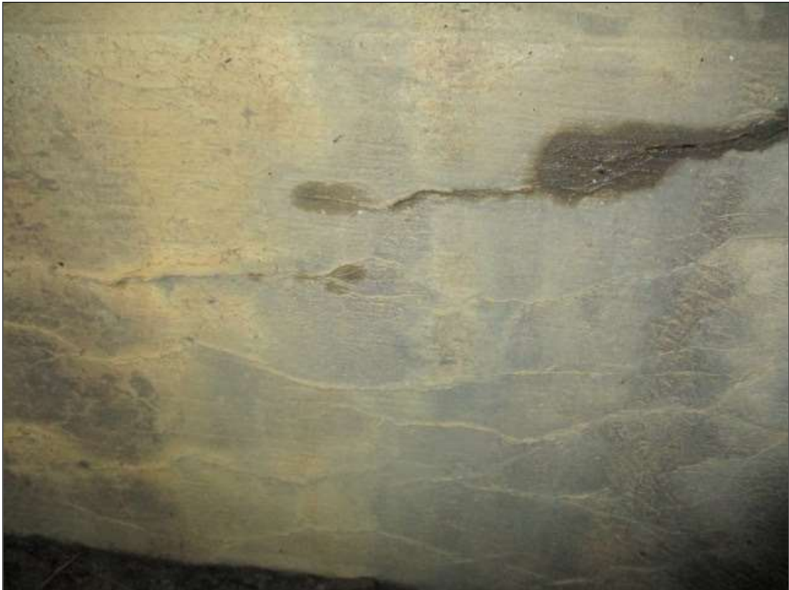
End Bent 1 Cap 1: 1/16" HORIZONTAL CRACKING THROUGHOUT
