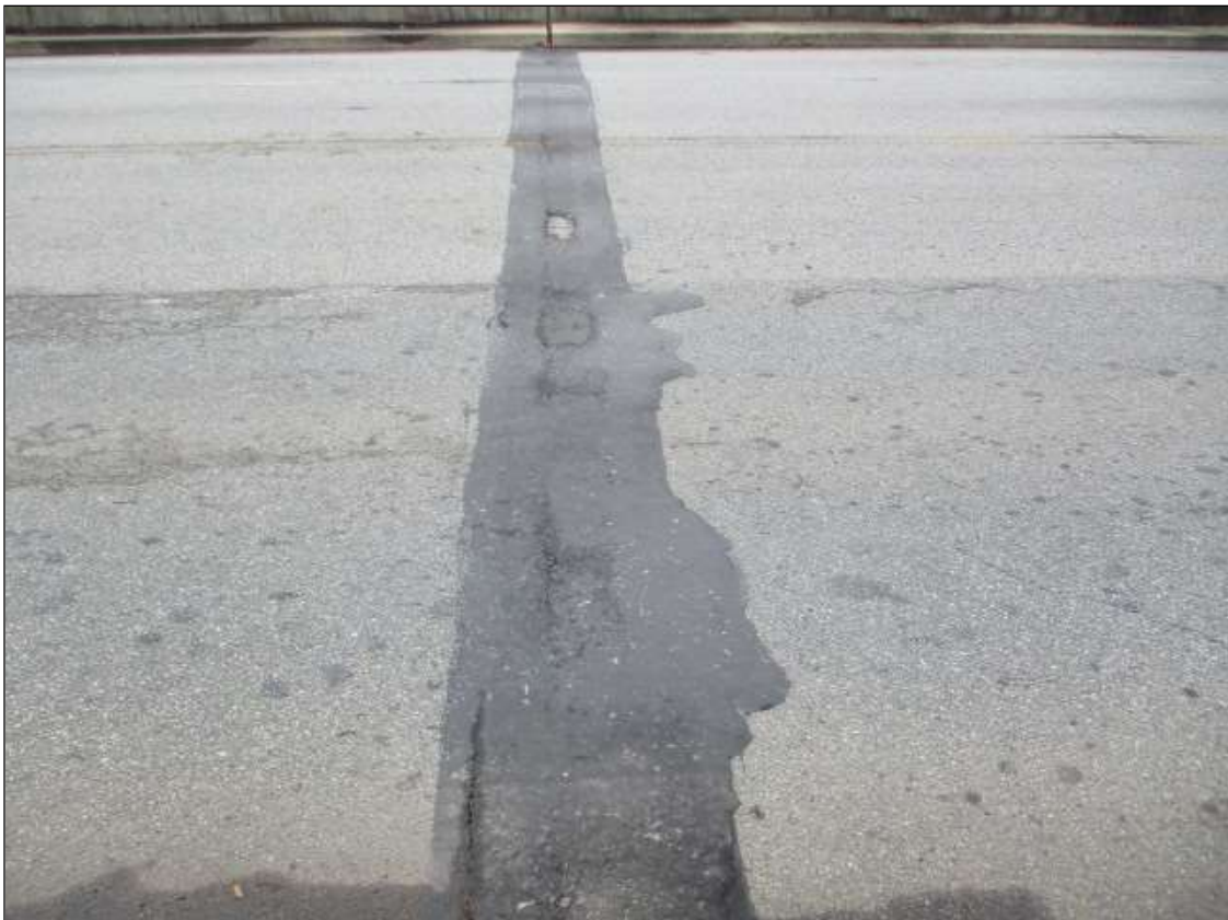
Span 2 Wearing Surface: PATCHED AREA OVER BENT 1
