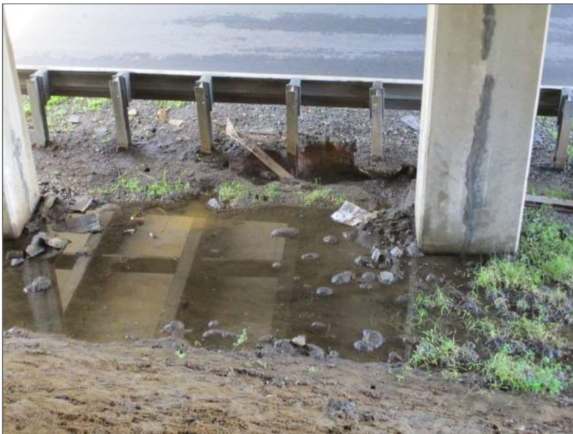
8' X 3' X 12" DEEP SINK HOLE UNDER BENT 2 BETWEEN COLUMNS 2 AND 3 AGAINST GUARDRAIL
