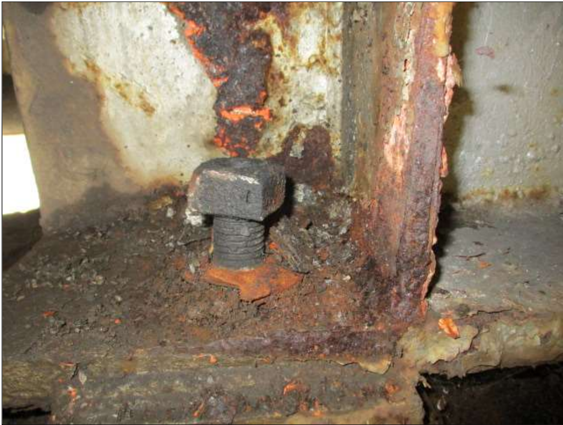
Span 1 Beam 8 Far Bearing: RAISED LEFT ANCHOR BOLT NUT BUT CANNOT BE MOVED BY HAND
