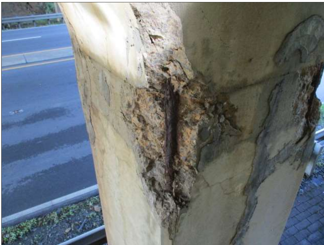
Bent 2 Pile 2: PAR: 3' X 10" X 11" SPALL WITH EXPOSED REBAR WITH SECTION LOSS ON SOUTHEAST CORNER AT TOP
