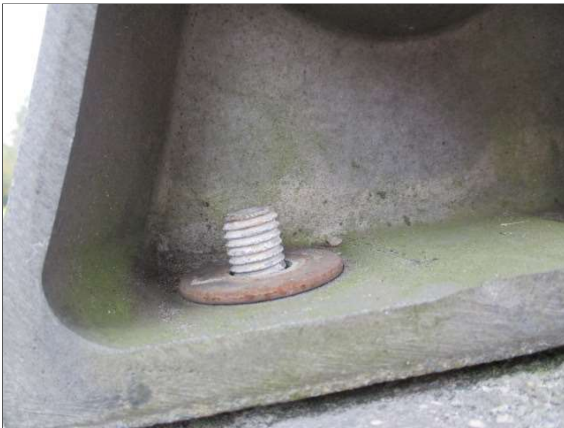
Span 2 Right Bridge Rail: PAR: MISSING BOLT NUT ON LAST POST IN SPAN
