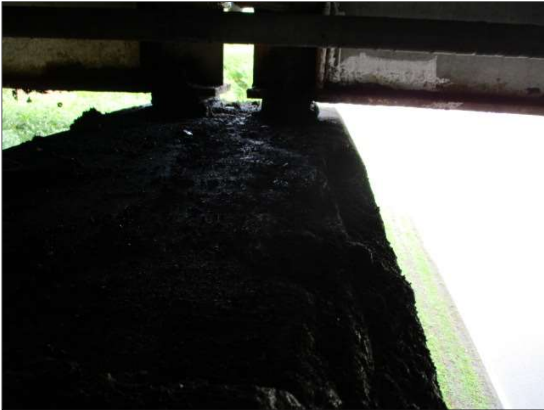
Bent 1 Cap 1: 4' X 6" X 5" SPALL WITH EXPOSED REBAR ON TOP OF CAP IN BAY 1 ON SPAN 2 SIDE
