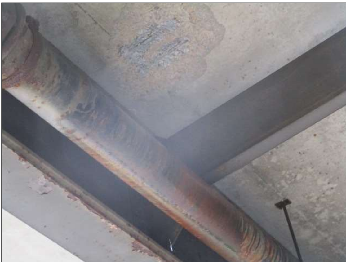
LEAKING UTILITY SECTION IN BAY 8 SPAN 2 OVER SOUTH BOUND LANES
