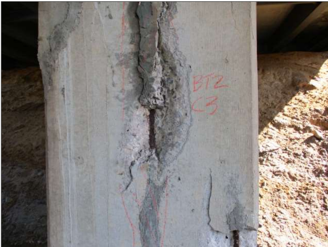
Bent 2 Pile 3: PAR: 30" X 11" X 2 1/2" SPALL WITH EXPOSED REBAR WITH SECTION LOSS ON WEST FACE
