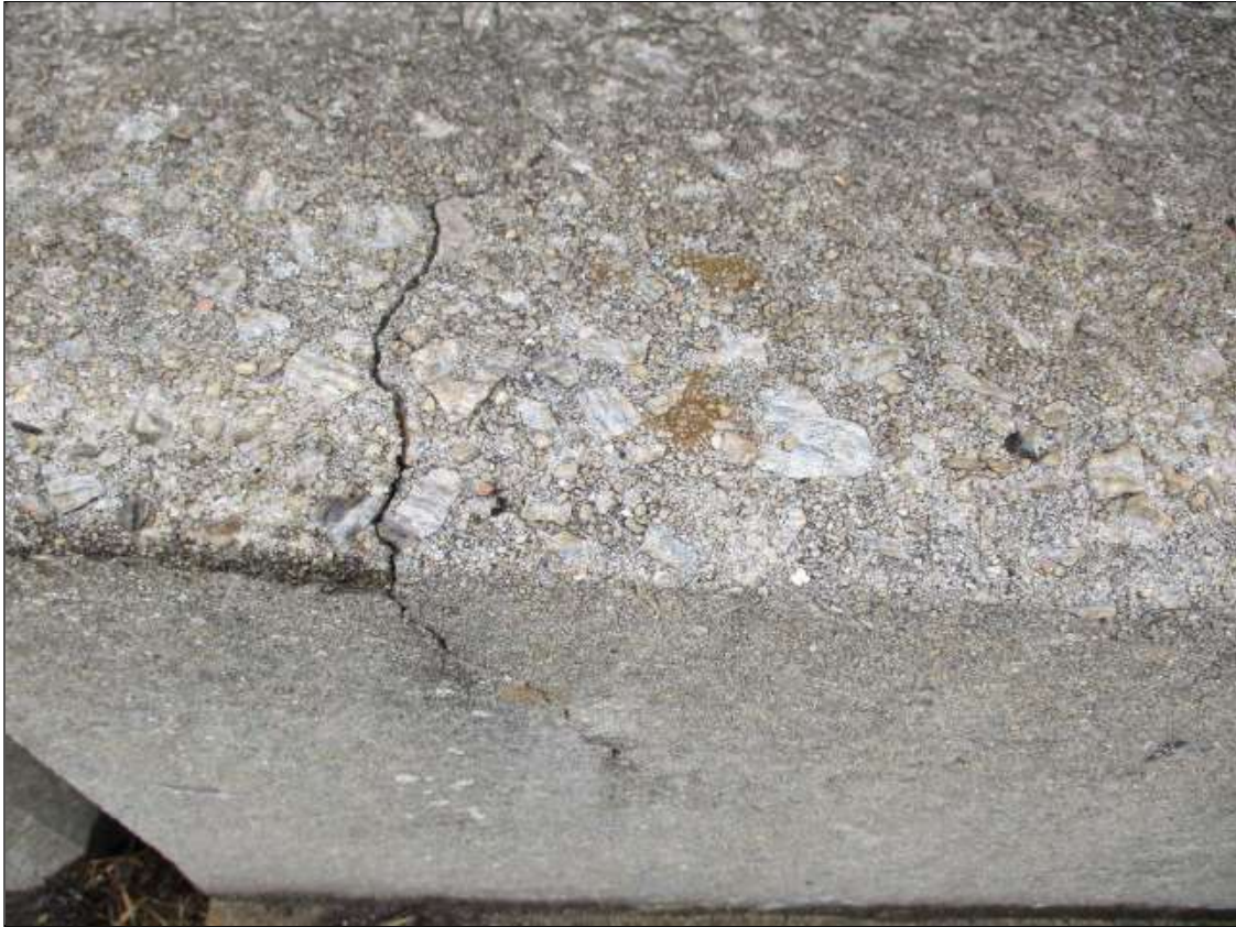
Span 1 Left Bridge Rail: 1/32" wide vertical cracks thru out the length of the rail
