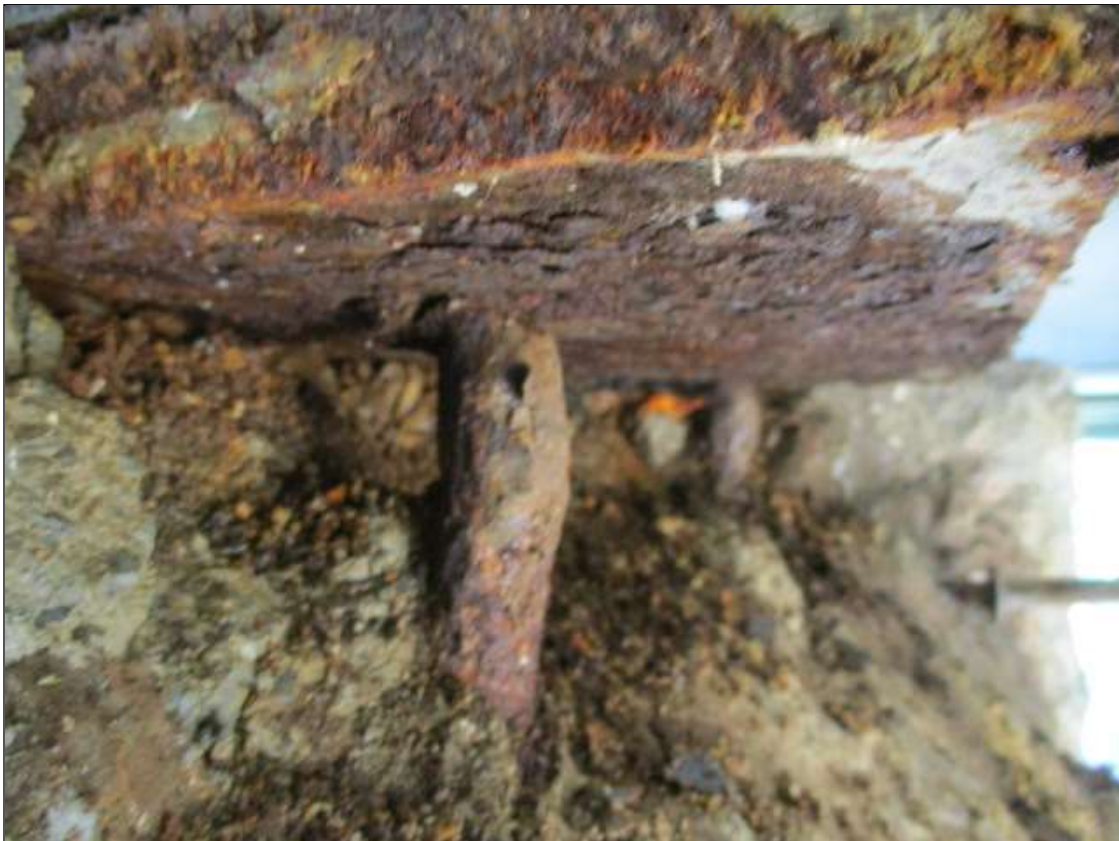
Span 3 Beam 7 - Beam 7 Near Bearing: PAR: SHEARED AND BENT BOLTS FROM BEARING TO CAP DUE TO LARGE SPALL ON CAP UNDER GIRDER
