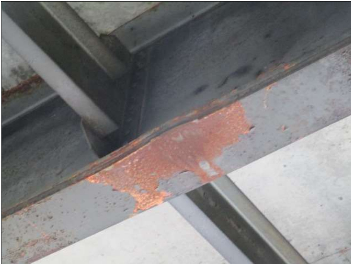
Span 2 Beam 7: PAR: at 21ft-7in from Bent 1 bearing, impact damage - bottom flange bent upward 2-1/8in, web bent 1-1/4in with gouge in bottom flange [1/8in deep], diaphragm 12in east of impact bent at bottom bolts
