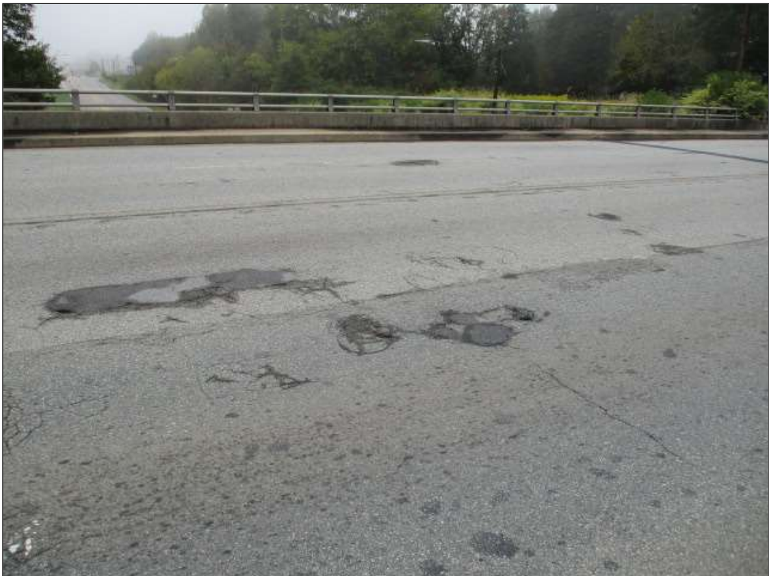
Span 2 Wearing Surface: MINOR POTHOLING IN TRAVEL LANES
