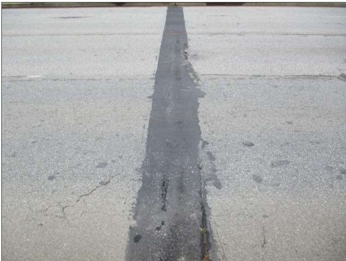
Span 3 Wearing Surface: PATCHED AREA OVER BENT 2
