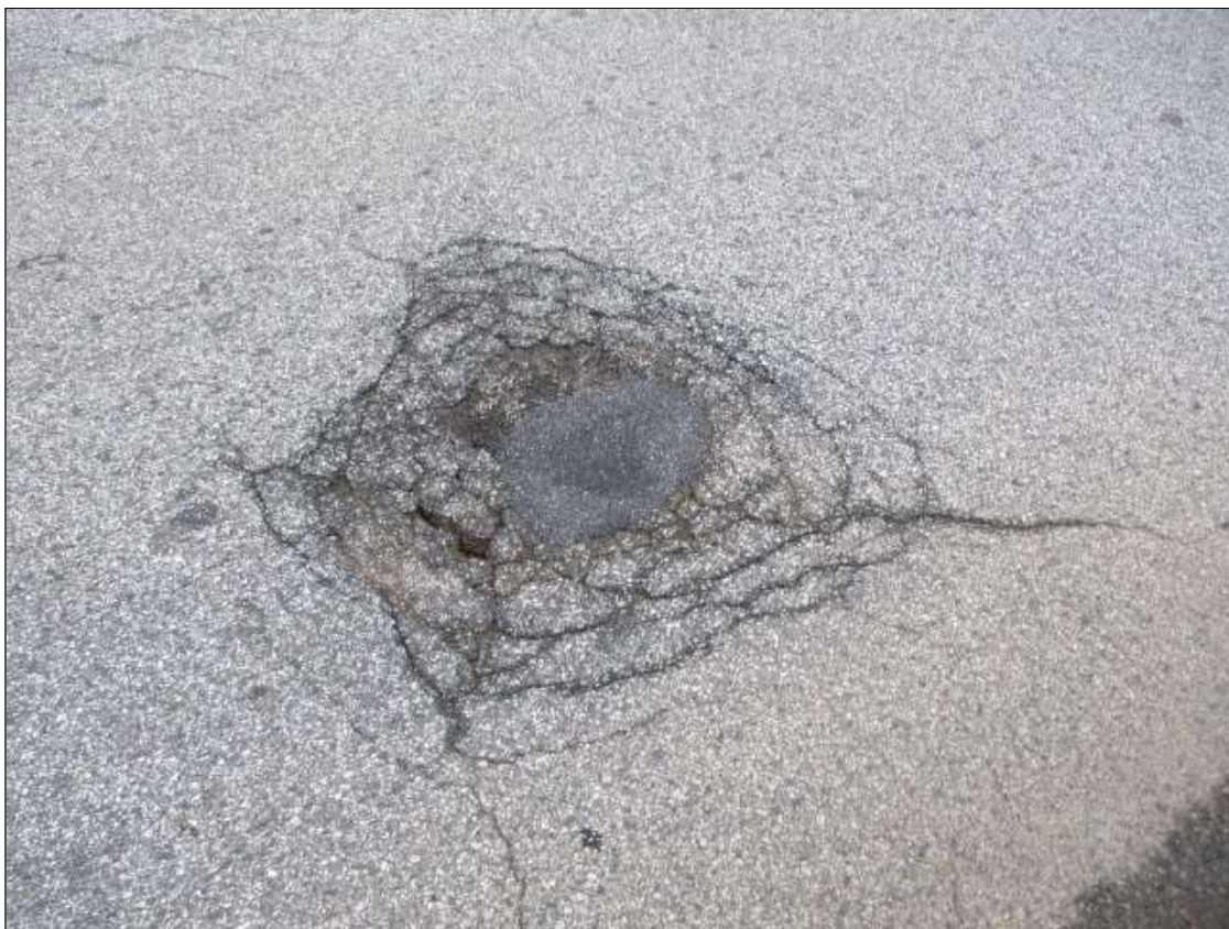
Span 1 Wearing Surface: 8 sq. ft. of sound patches thru out the top of the wearing surface
