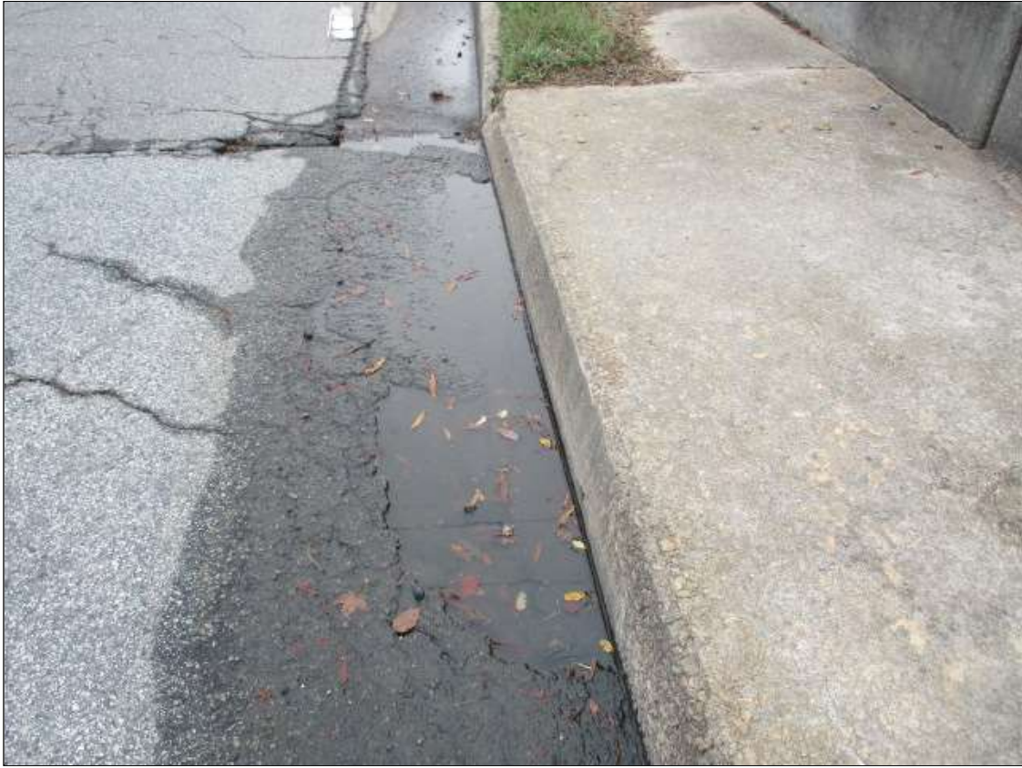
Span 3 Wearing Surface: 8' X 16" X 1 1/2" DEEP POTHOLE IN RIGHT EAST BOUND LANE AT END BENT 2
