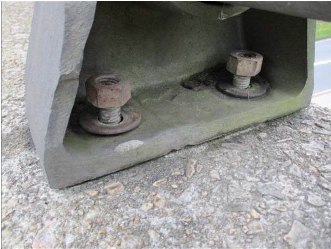
Span 2 Left Bridge Rail: RAISED ANCHOR NUTS ON 2ND TO LAST RAIL POST
