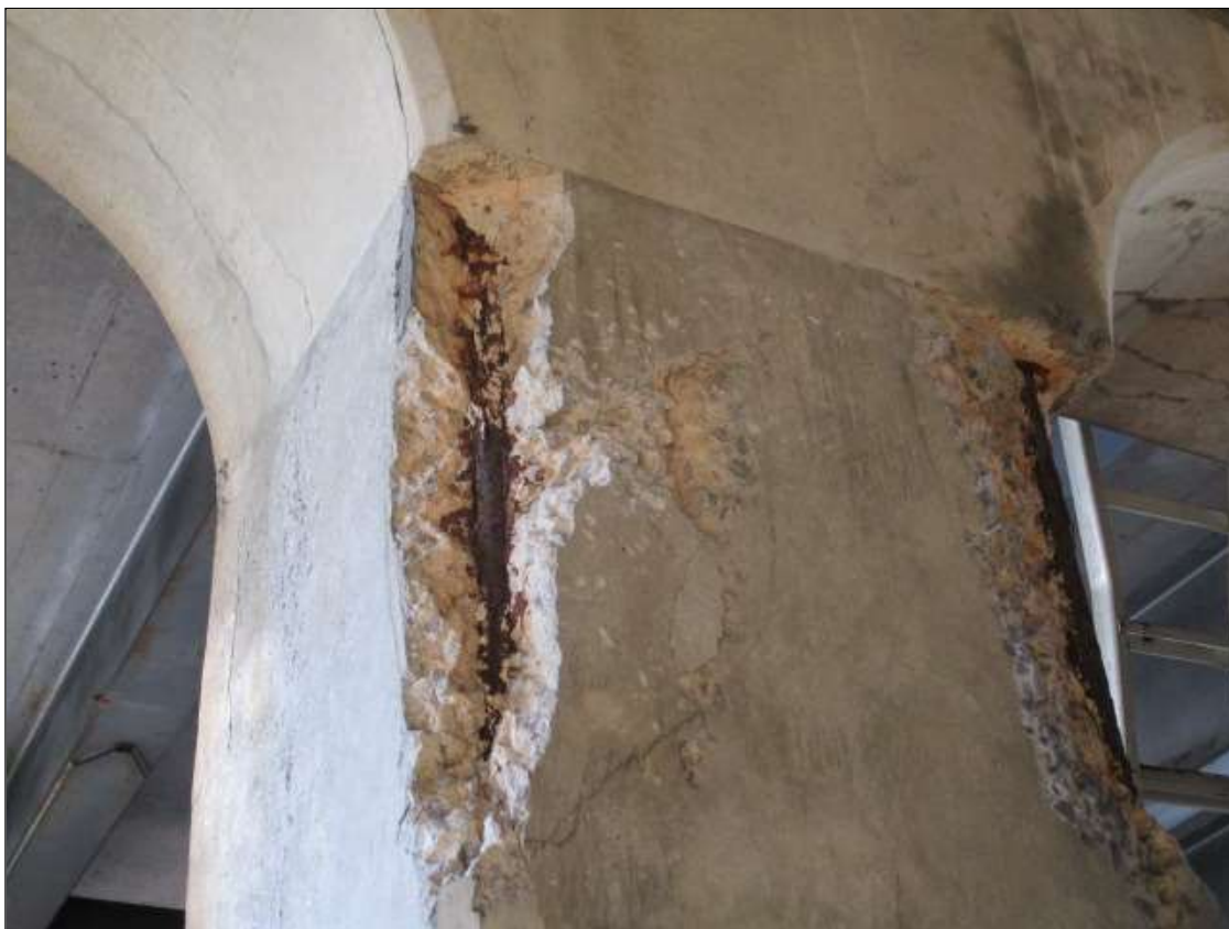
Bent 2 Pile 3: PAR: 3' X 6" X 6" SPALL WITH EXPOSED REBAR WITH SECTION LOSS ON SOUTHEAST CORNER
