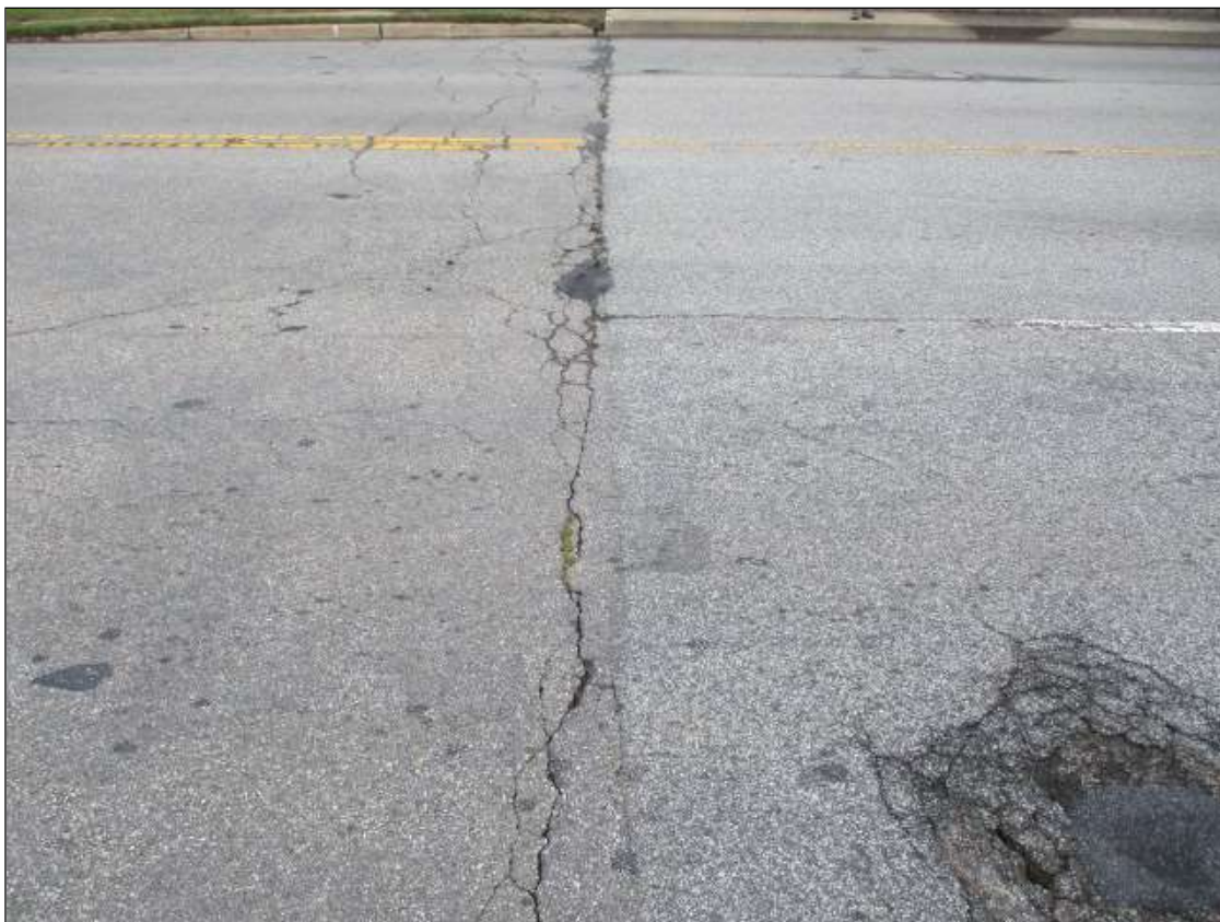
Span 1 Wearing Surface: 1" TRANSVERSE CRACK OVER END BENT 1
