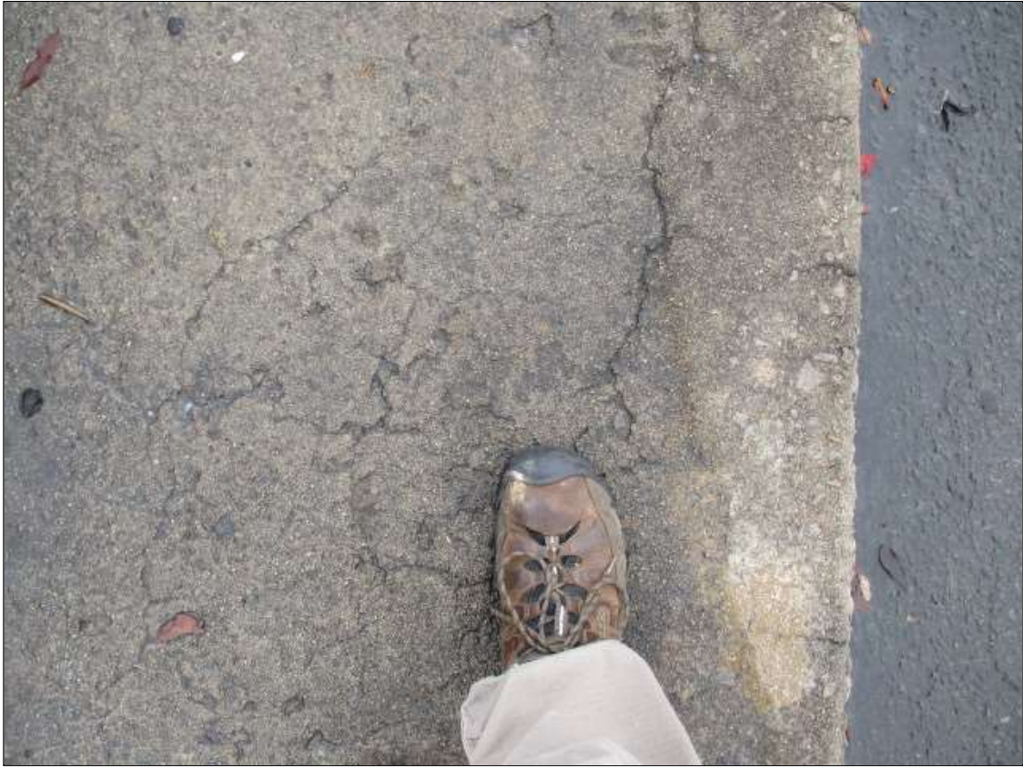
1/32" MAP CRACKING ALONG SIDEWALKS
