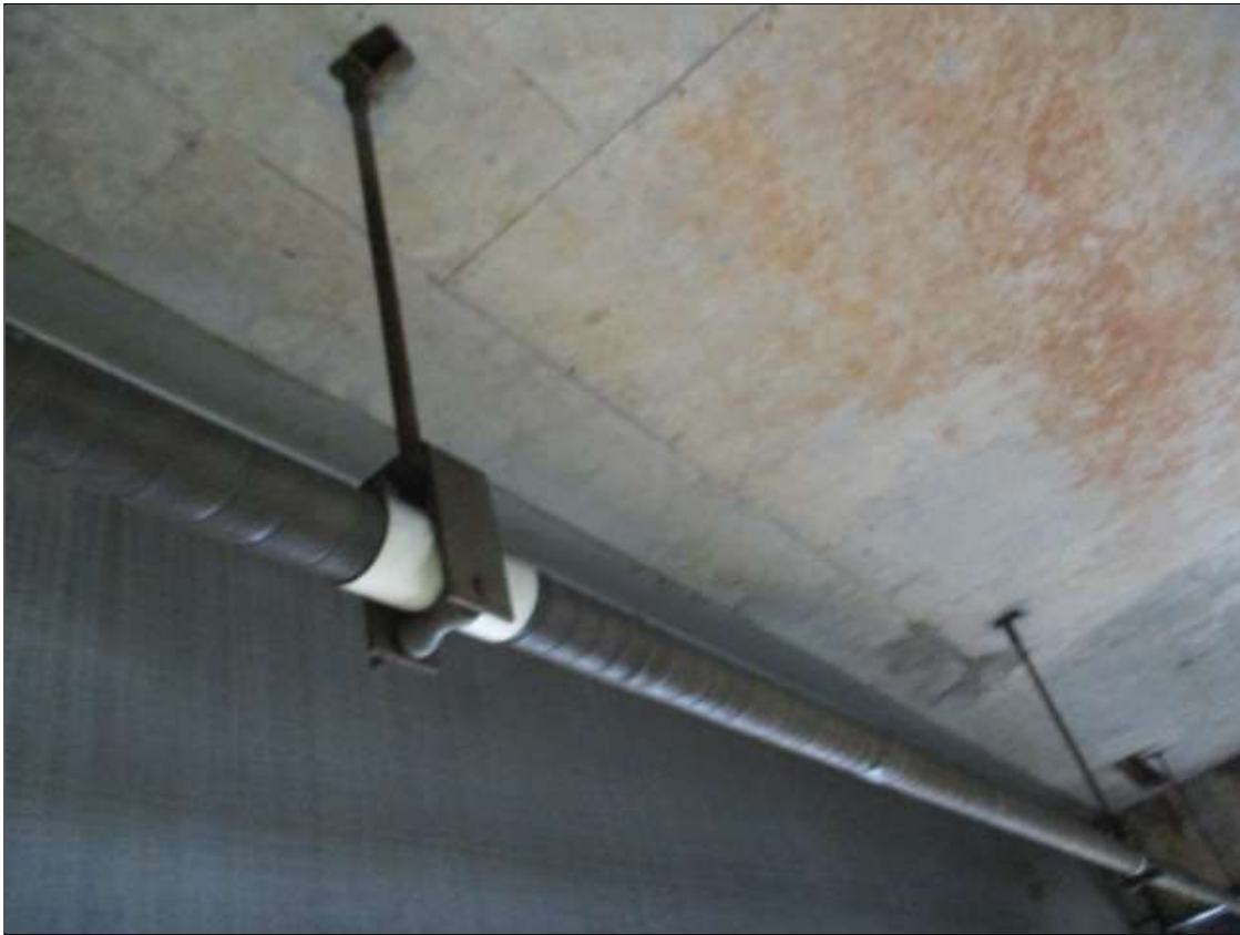
UTILITY IN BAY 1
