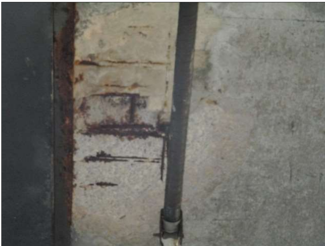
Span 2 Deck: PAR: 3' DIAMETER X 2" DEEP SPALL WITH EXPOSED REBAR WITH SECTION LOSS IN BAY 1 AT 2ND UTILITY HANGER
