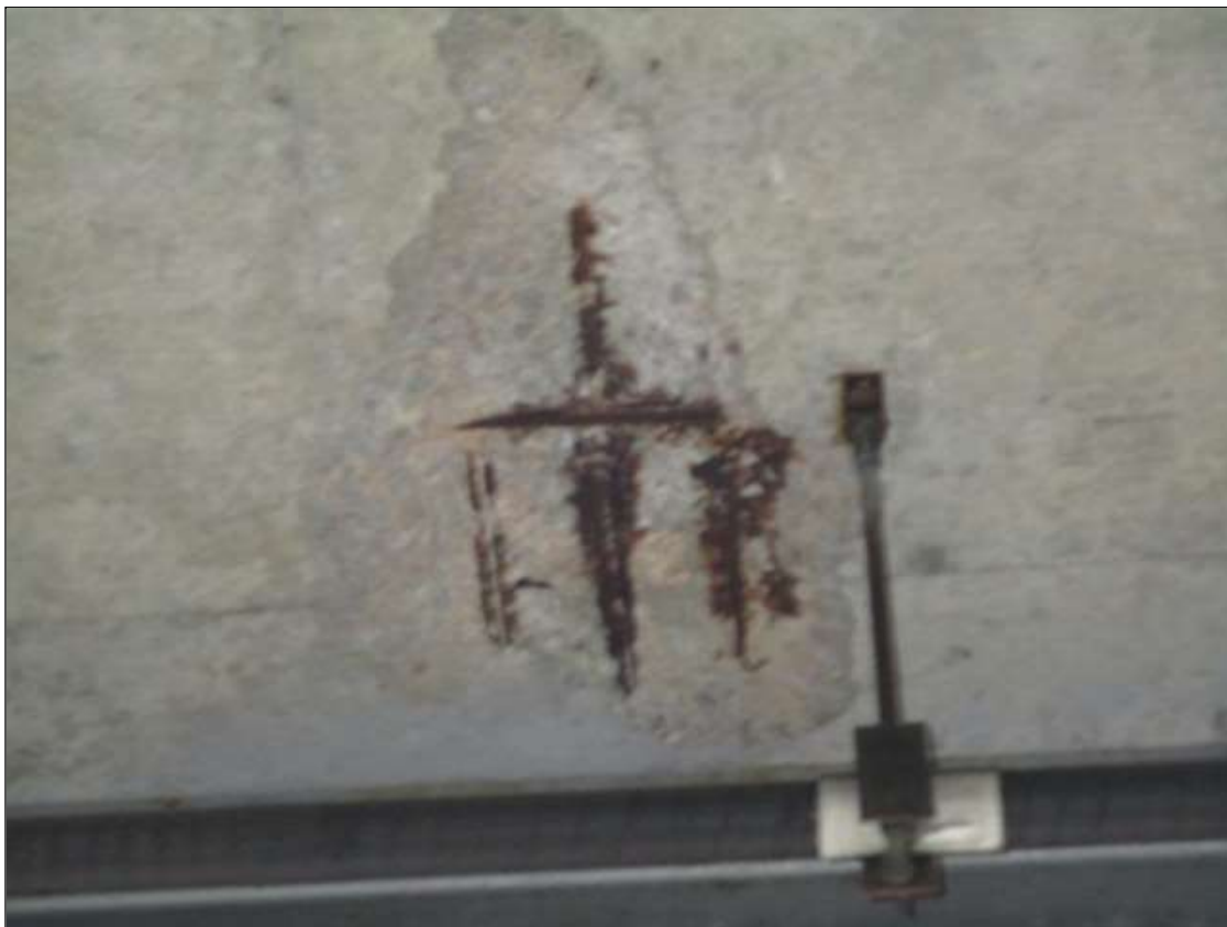
Span 2 Deck: PAR: 30" X 20" X 2" DEEP SPALL WITH EXPOSED REBAR WITH SECTION LOSS IN BAY 1 AT 5TH UTILITY HANGER
