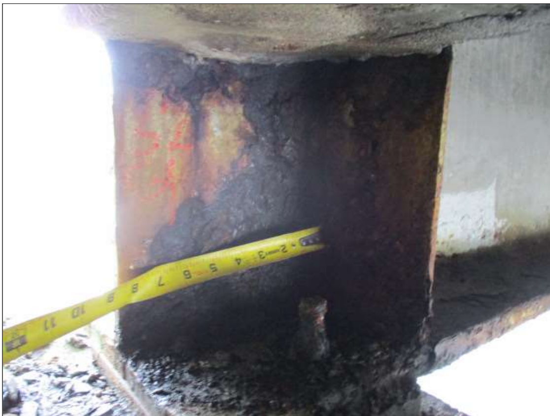
Span 2 Beam 1: PAR: 3/8" REMAINING (1/4" SECTION LOSS) ON FULL HEIGHT OF WEB UNDER DIAPHRAGM FOR 8" LONG AT BENT 1
