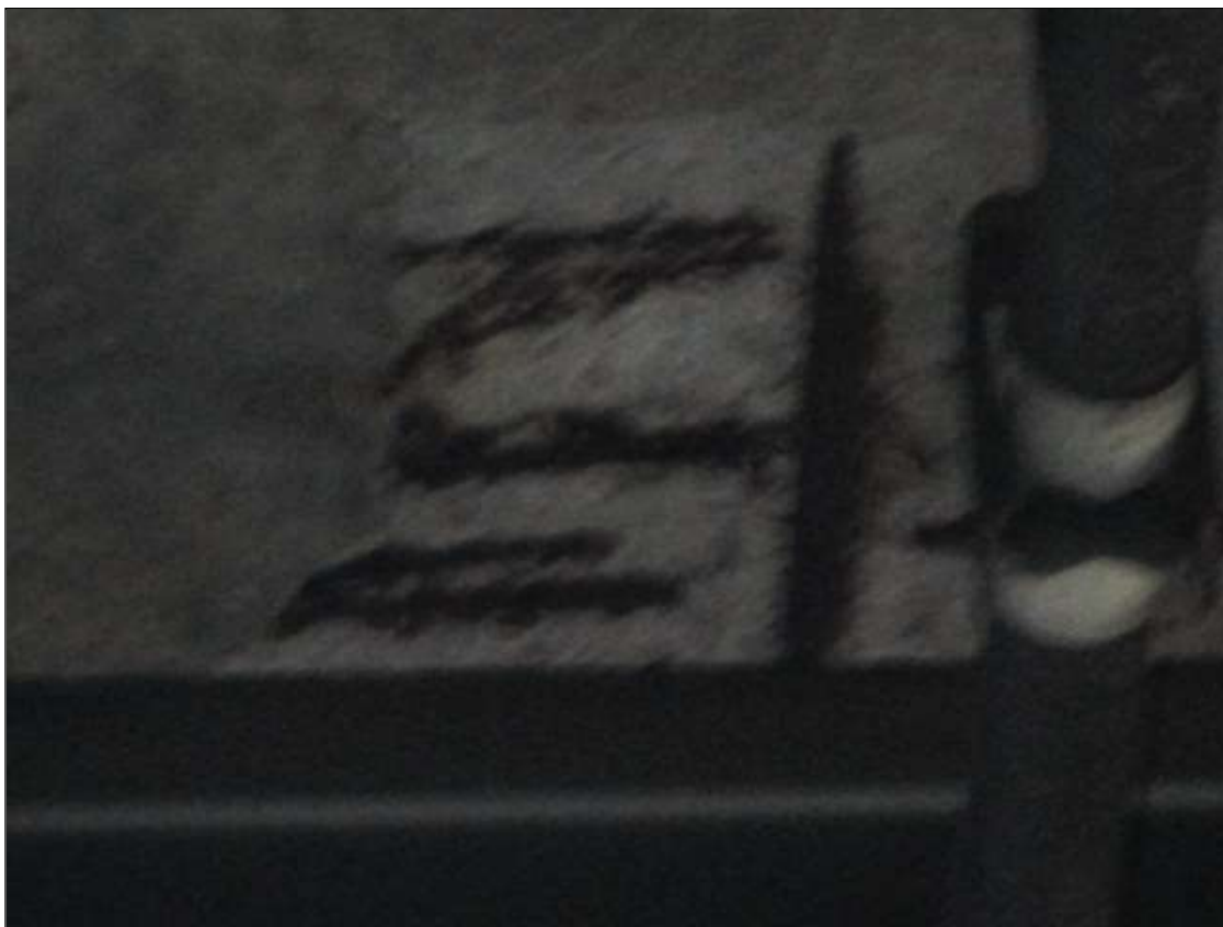
Span 2 Deck: PAR: 18" X 12" X 2" DEEP SPALL WITH EXPOSED REBAR WITH SECTION LOSS IN BAY 1 OVER FIRST DIAPHRAGM
