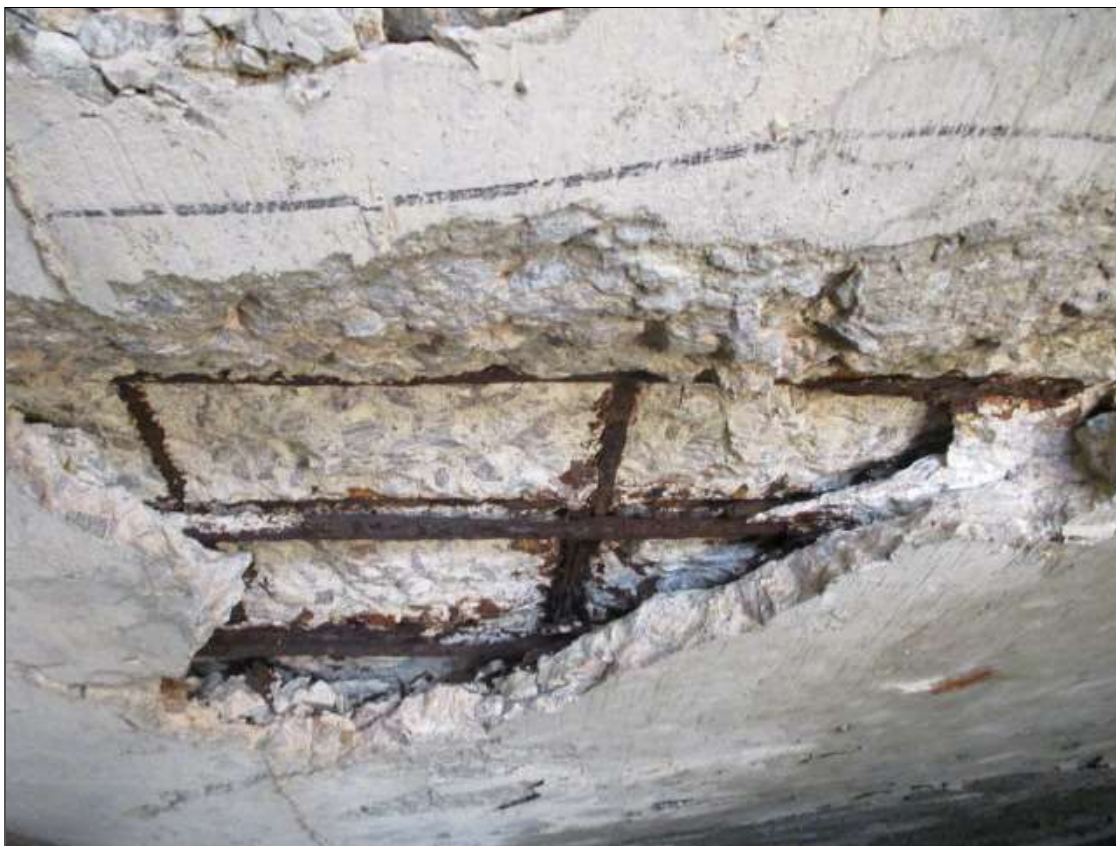
Span 3 Deck: PAR: 30" X 24" X 3" DEEP SPALL WITH EXPOSED REBAR WITH SECTION LOSS IN BAY 8 AT 8' FROM END BENT 2
