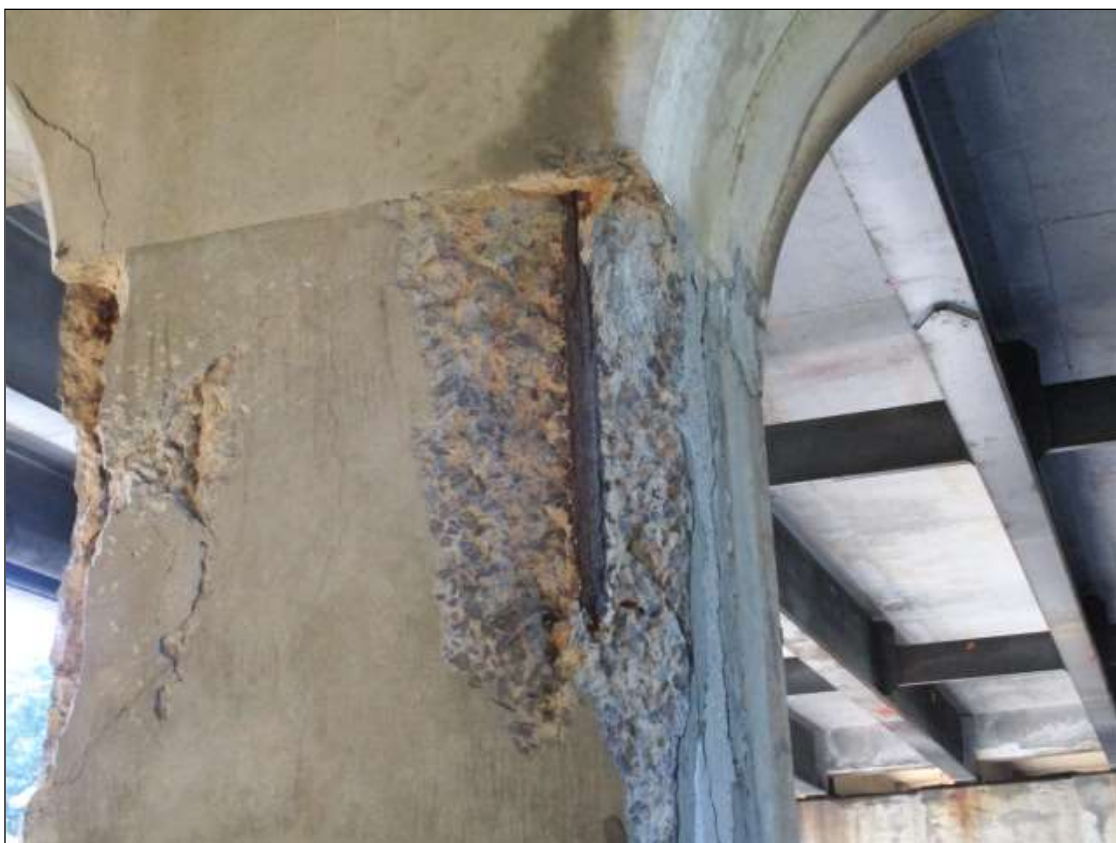
Bent 2 Pile 3: PAR: 3' X 15" X 12" SPALL WITH EXPOSED REBAR WITH SECTION LOSS ON NORTHEAST CORNER
