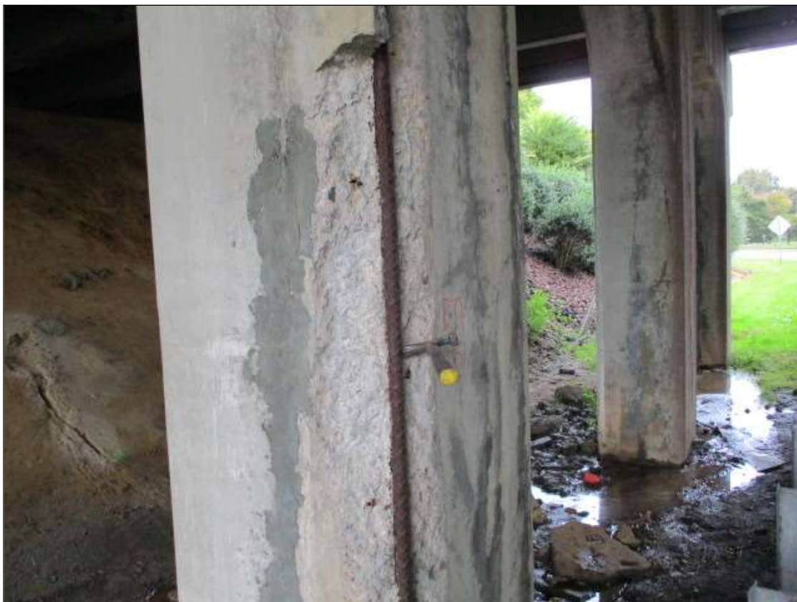
Bent 1 Pile 3: PAR: 9' X 8" X 8" SPALL WITH EXPOSED REBAR WITH SECTION LOSS ON SOUTHEAST CORNER
