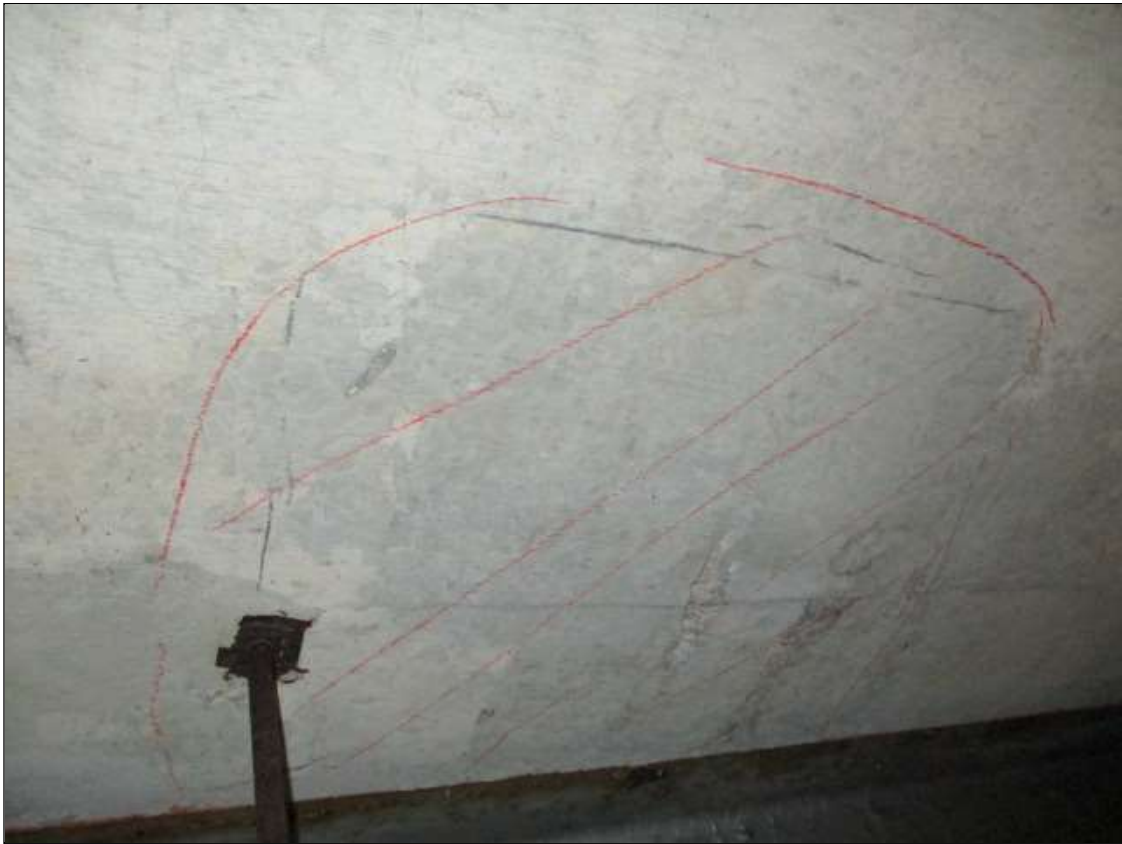
Span 1 Deck: 30" X 24" DELAMINATION IN BAY 8 NEAR END BENT 1
