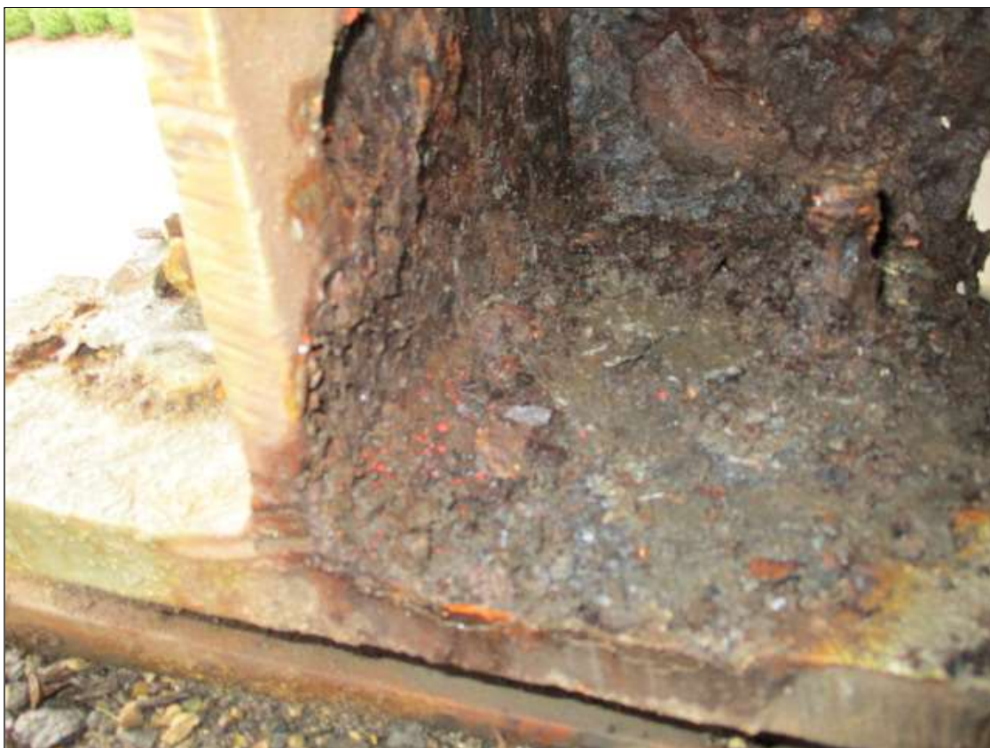
Span 2 Beam 1 - Beam 1 Near Bearing: PAR: MISSING RIGHT ANCHOR BOLT NUT
