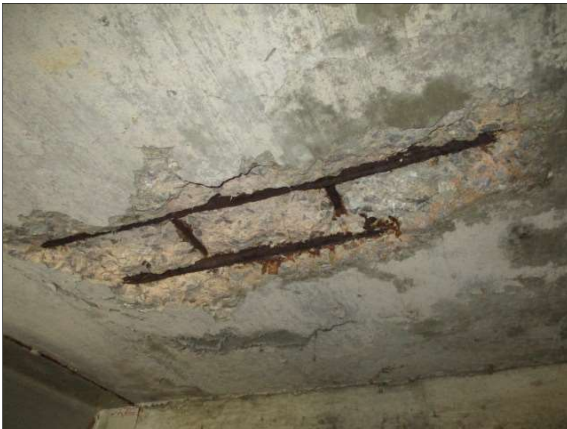
Span 3 Deck: PAR: 30" X 15" X 2 1/2" DEEP SPALL WITH EXPOSED REBAR WITH SECTION LOSS IN BAY 7 AT 2' FROM END BENT 2
