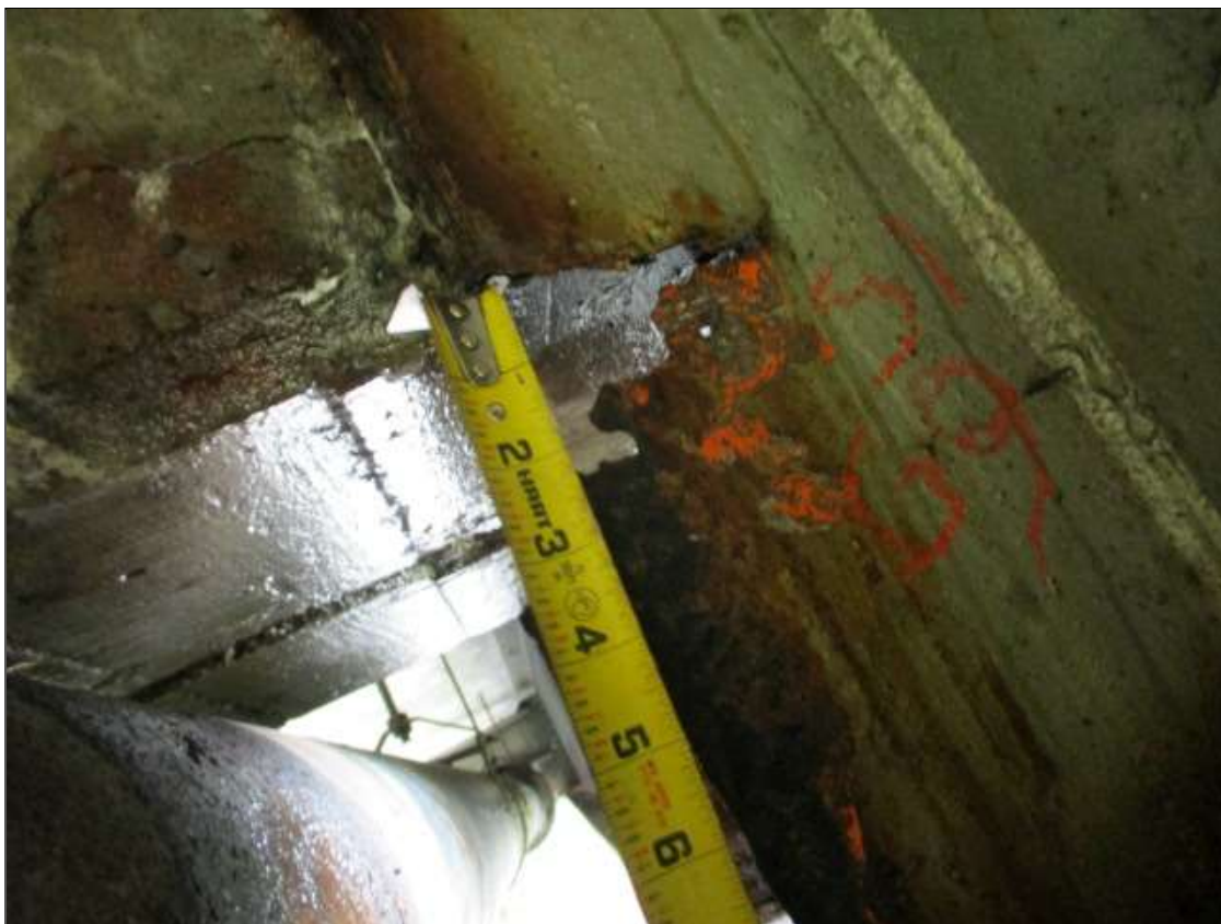
Span 1 Beam 9: PAR: 2 1/2" X 3 1/2" HOLE IN LEFT STIFFENER AT DIAPHRAGM AT BENT 1
