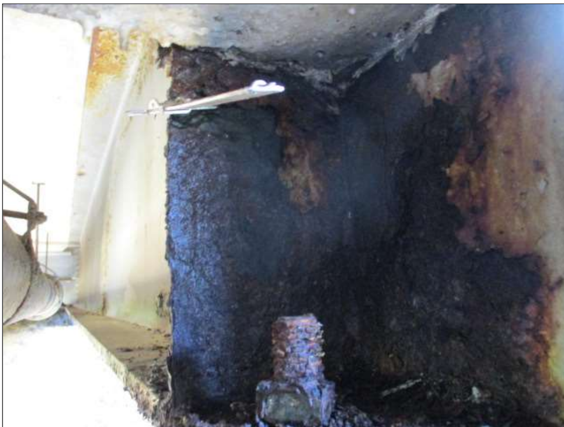
Span 3 Beam 9: PAR: 3/16" REMAINING (3/16" SECTION LOSS) IN LEFT STIFFENER FOR FULL HEIGHT AT BENT 2
