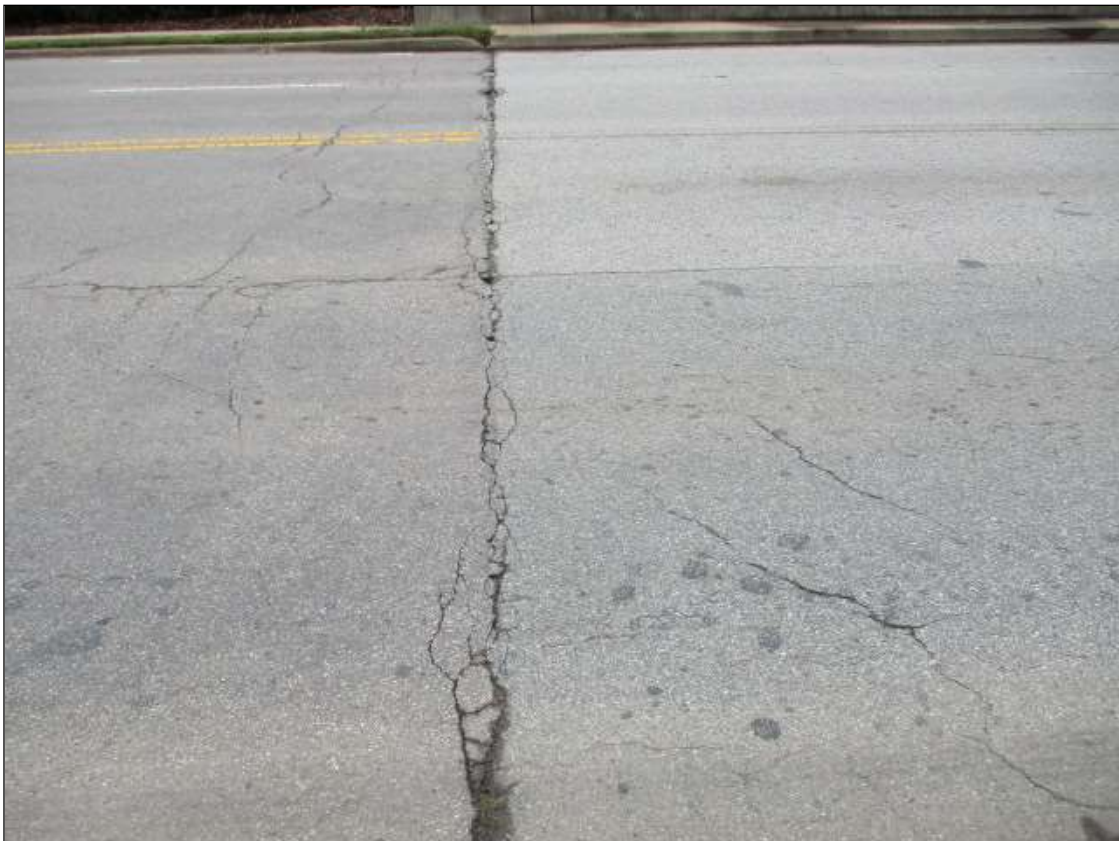
Span 3 Wearing Surface: 1" TRANSVERSE CRACK OVER END BENT 2
