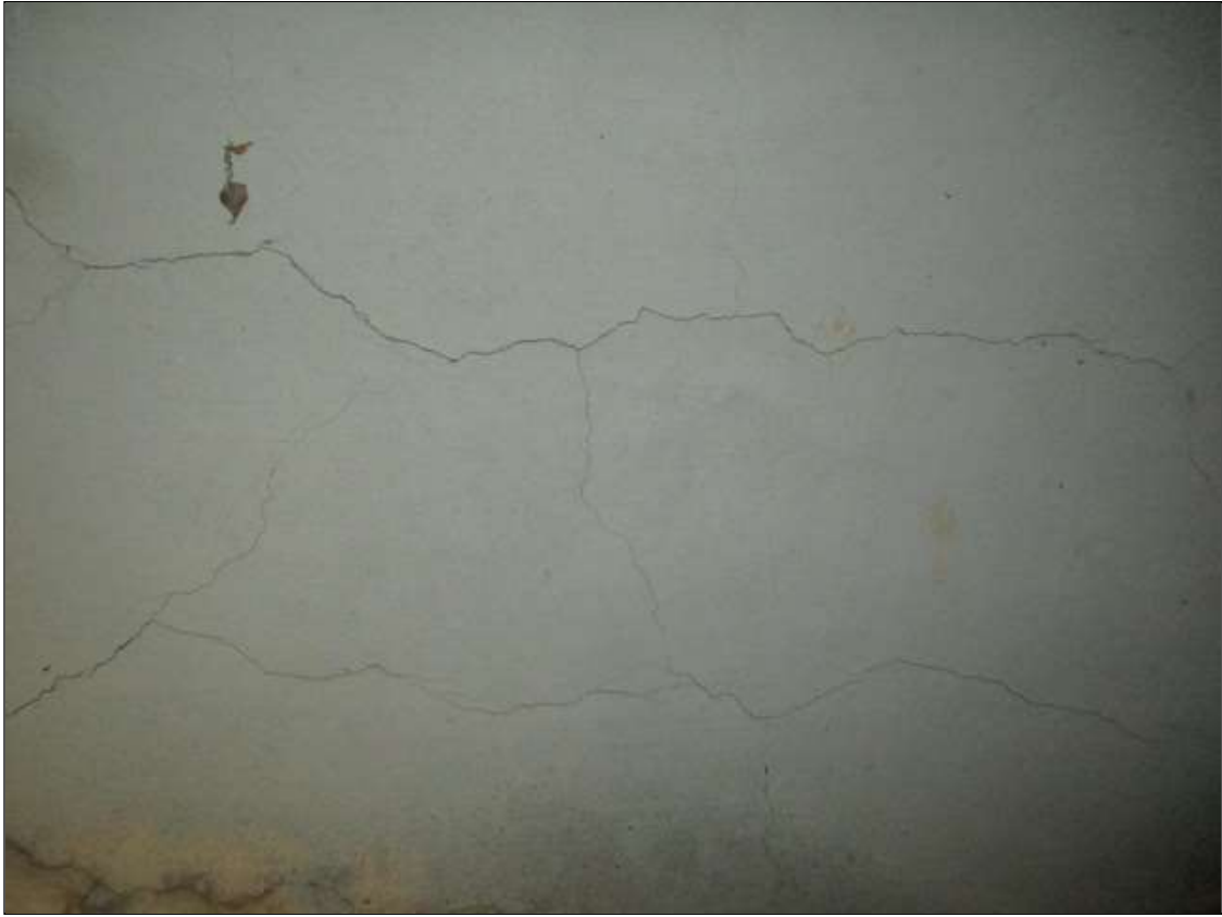
End Bent 1 Abutment: 1/32" MAP CRACKING THROUGHOUT BACKWALL
