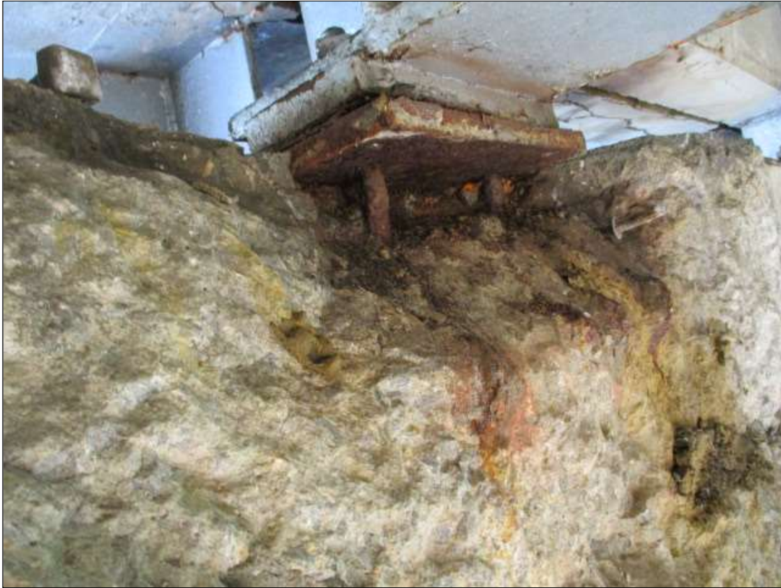
Bent 2 Cap 1: PAR: 51" X 18" X 11" DEEP SPALL WITH EXPOSED REBAR WITH SECTION LOSS UNDER GIRDER 7 SPAN 3 WITH UP TO 6.5" DEEP LOSS OF BEARING
