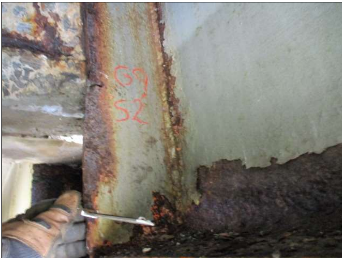
Span 2 Beam 9: PAR: 3/4" X 3/4" HOLE IN LEFT STIFFENER AT DIAPHRAGM AT BENT 2
