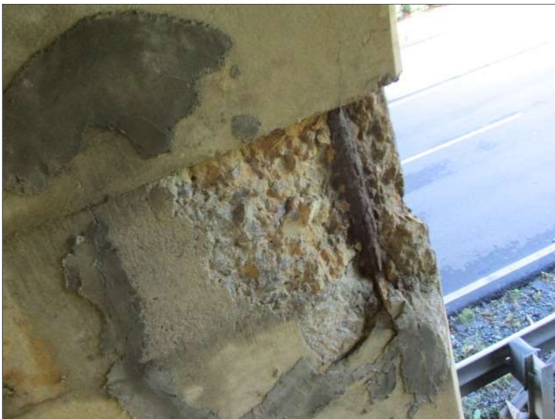
Bent 2 Pile 2: PAR: 16" X 15" X 4" SPALL WITH EXPOSED REBAR WITH SECTION LOSS ON NORTHEAST CORNER AT TOP
