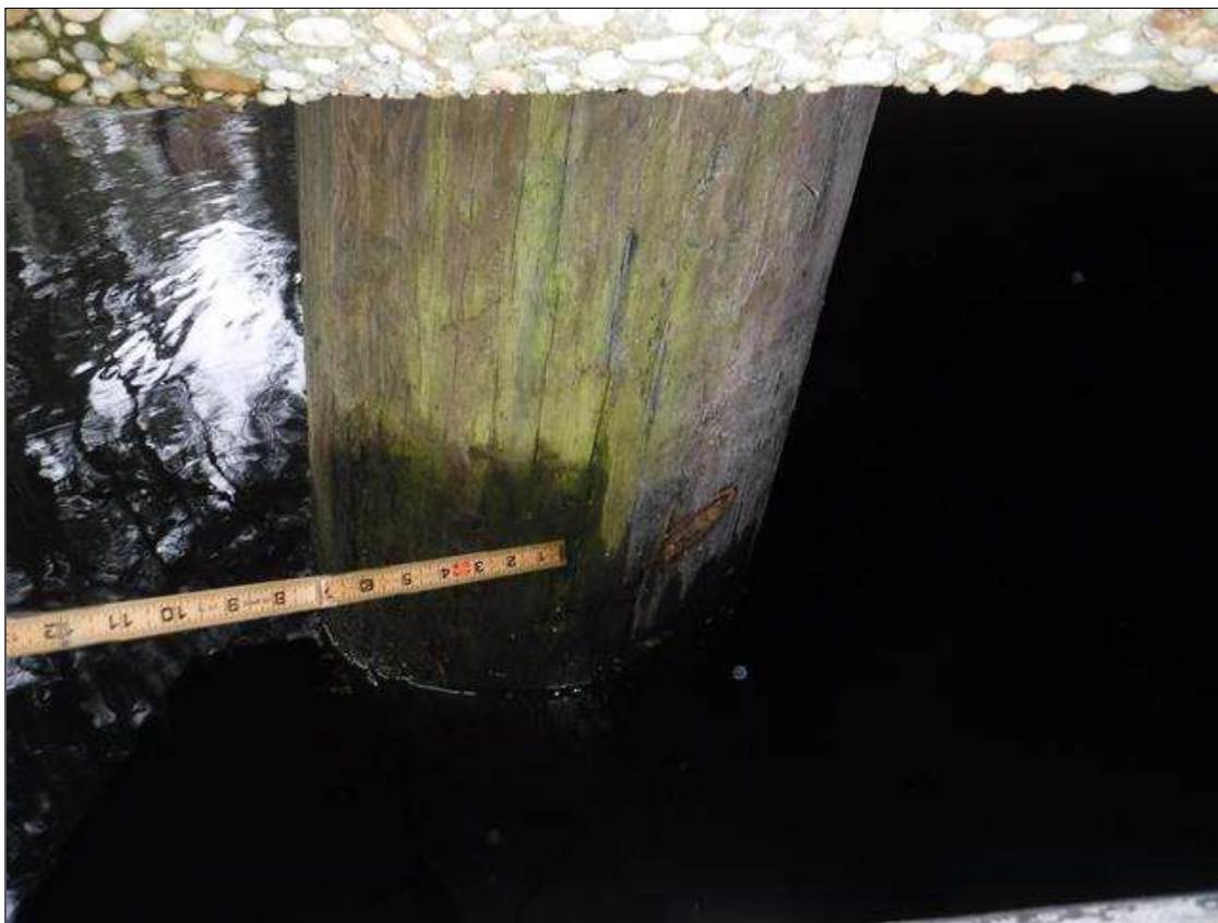
Decay, (1/2" deep x 12" x 12".)
