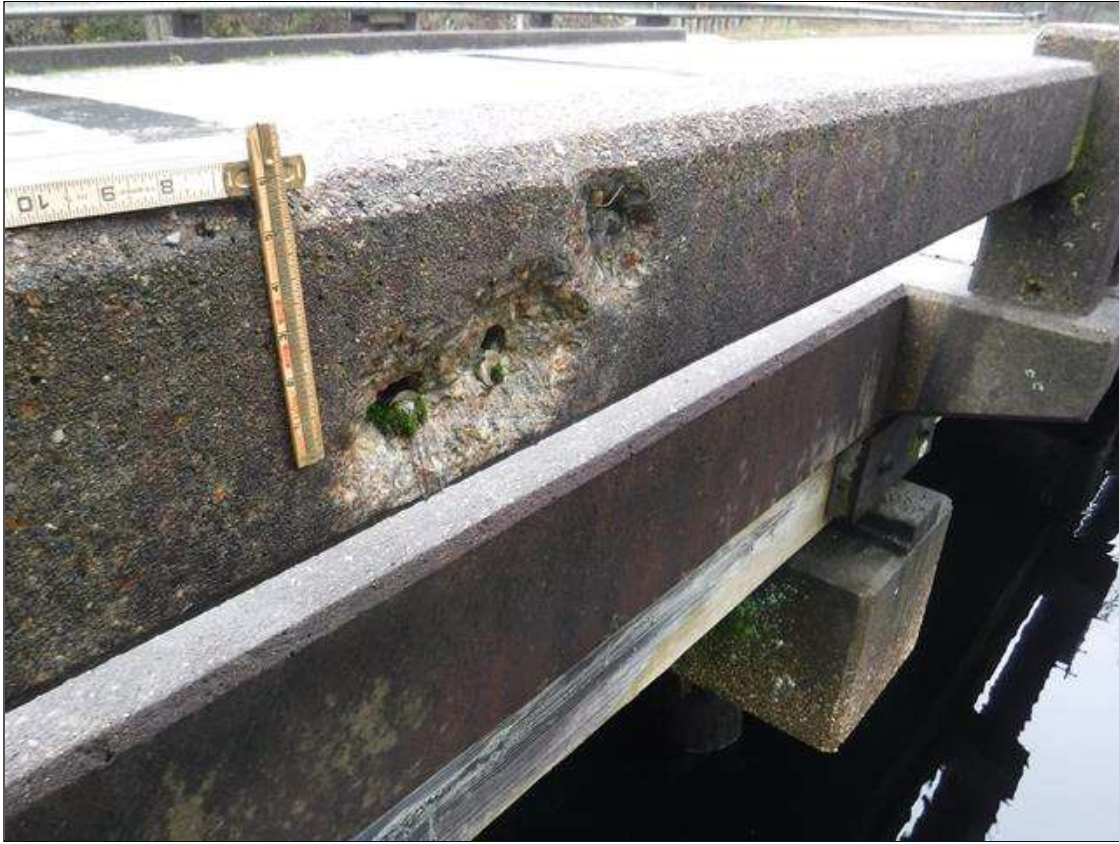
SPALL NO EXPOSED STEEL, (15" X 4" X 1") EXTERIOR SIDE OF RAIL AT PREVIOUS GUARDRAIL CONNECTION.
