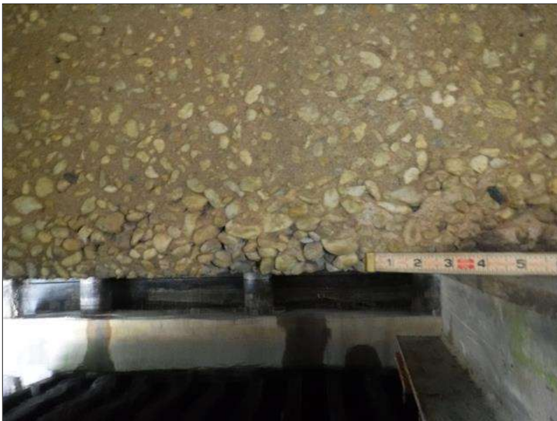
Bent 2 Cap 1: ABRASION UP TO 1" DEEP, EXPOSING AGGREGATE, 12" HIGH
