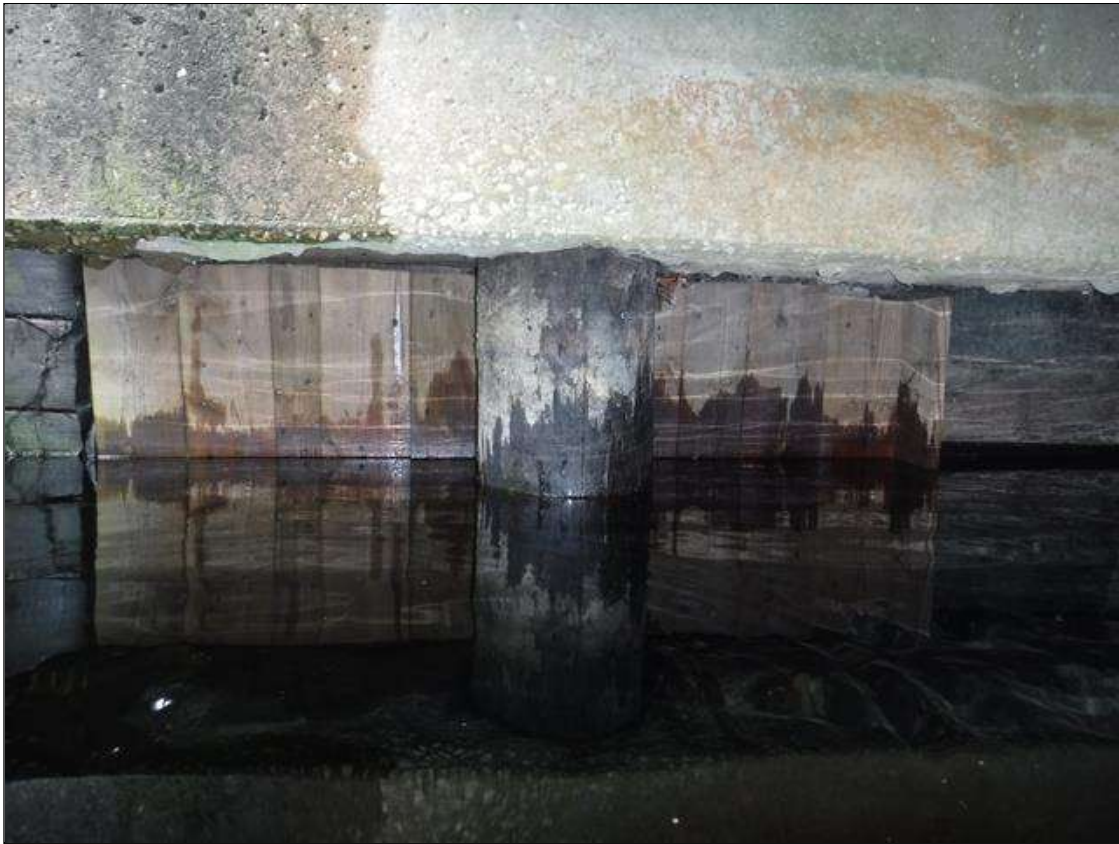
BOTH SIDES OF PILE 4, TIMBER BULKHEAD BOARDS REPLACED (PREVIOUS REPAIR) (6' LONG)
