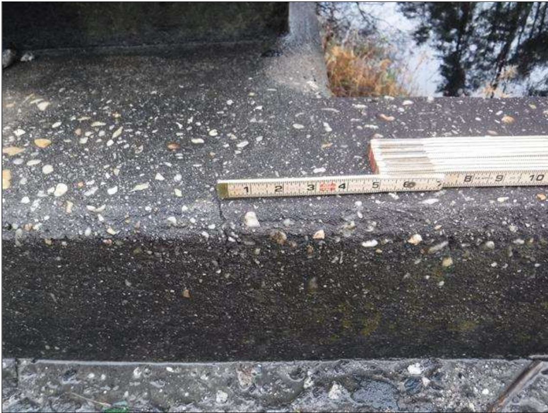
HAIRLINE TRANSVERSE CRACKING SCATTERED ALONG CURBS
