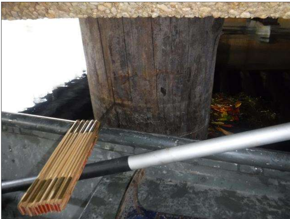
CHECKS ALONG THE PILES UP TO .066" WIDE
