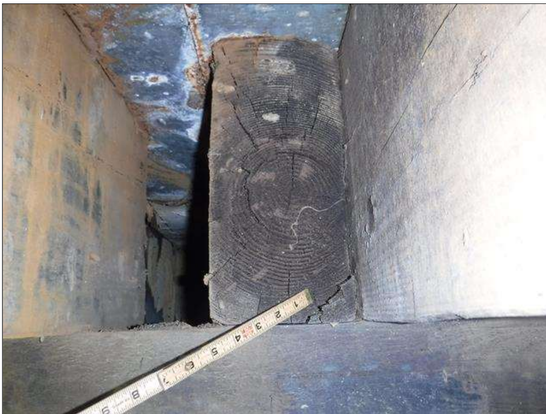
Span 1 Beam 7: 16" X 3" X 3" AREA OF DELAMINATION IN BOTTOM LEFT CORNER OF JOIST AT BENT 1
