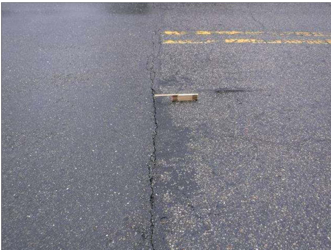
Span 1 Wearing Surface: UP TO 1/4" TRANSVERSE CRACK ALONG END BENT 1 FILL FACE
