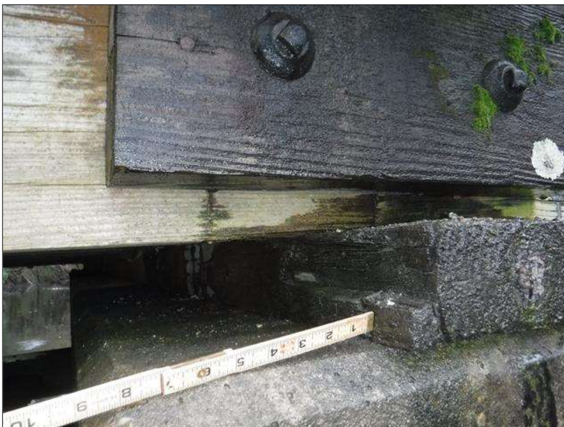
Timber Crown Strip at right end of cap, decay / Section Loss (10" long x 2-1/2" x 1-1/2".)
