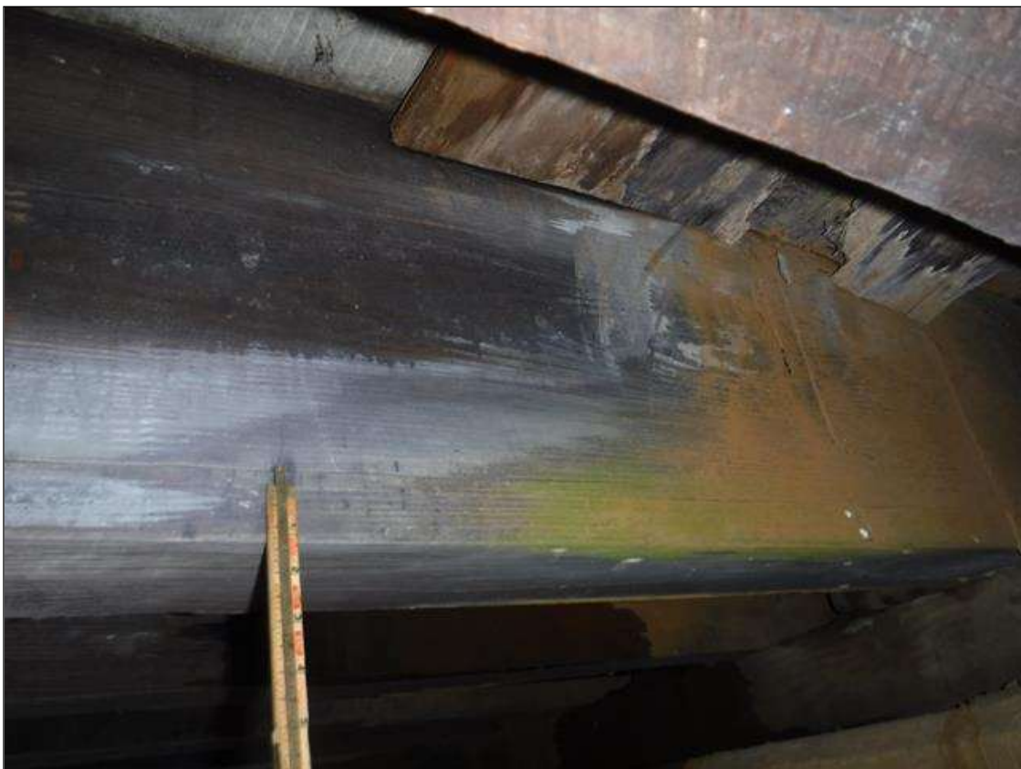
CHECKS ALONG THE JOIST UP TO .062" WIDE
