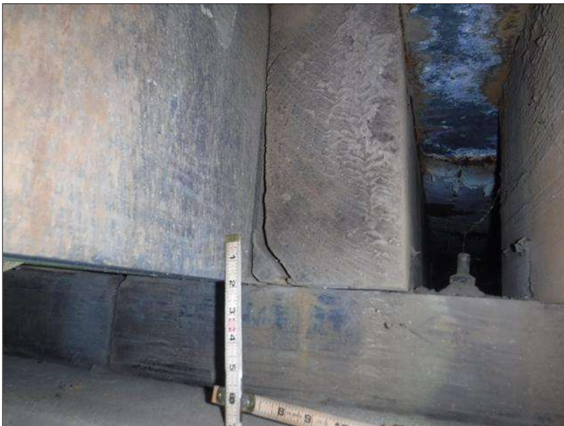
Span 3 Beam 10: 12" X 3" X 2" SPLIT IN BOTTOM LEFT CORNER OF JOIST AT BENT 2
