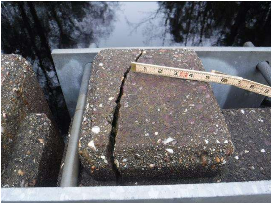
POST #3 CRACKED AREA (UP TO 3/8" WIDE X FULL WIDTH)
