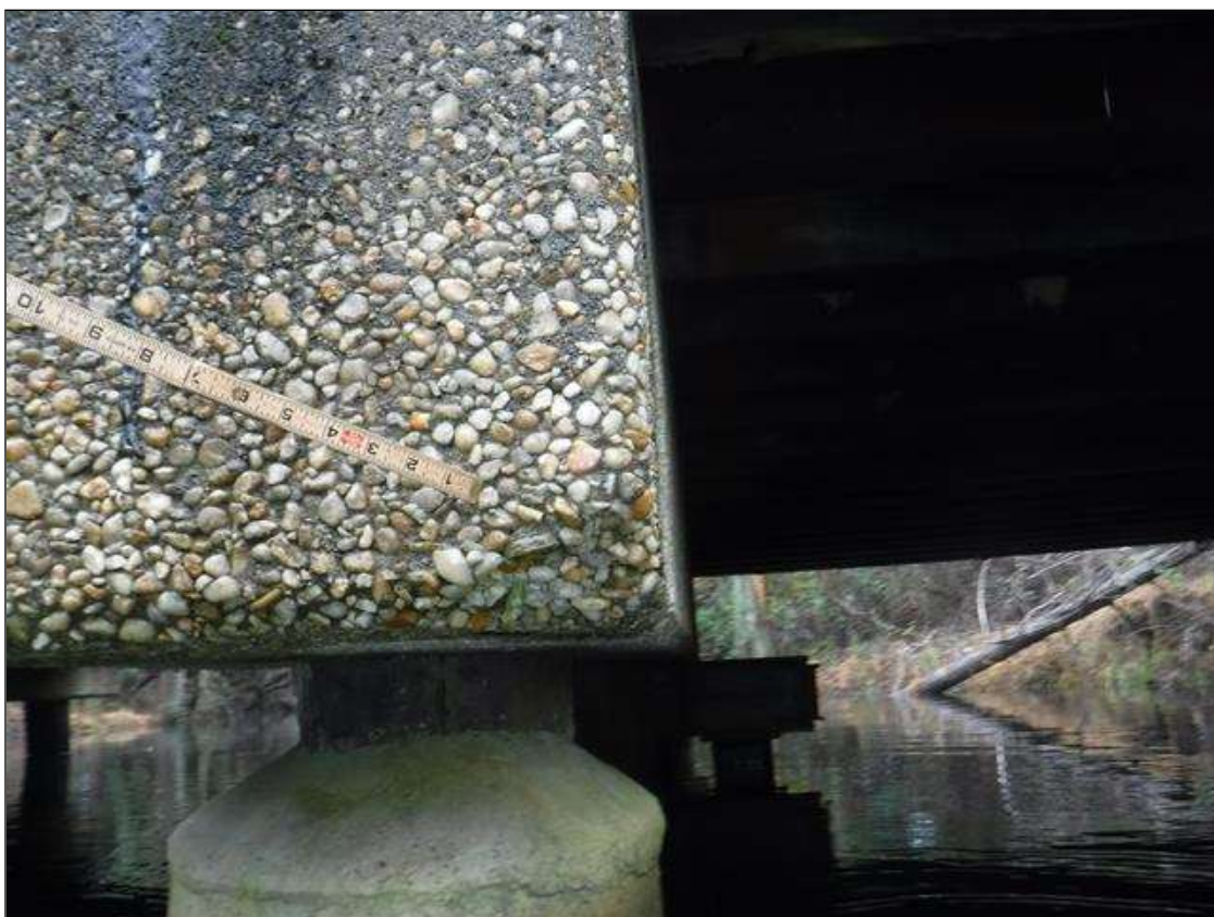
EAST END AT LOWER CORNER SPALLED AREA, no exposed steel, (5"LONG X 6"WIDE X 6"HIGH)
