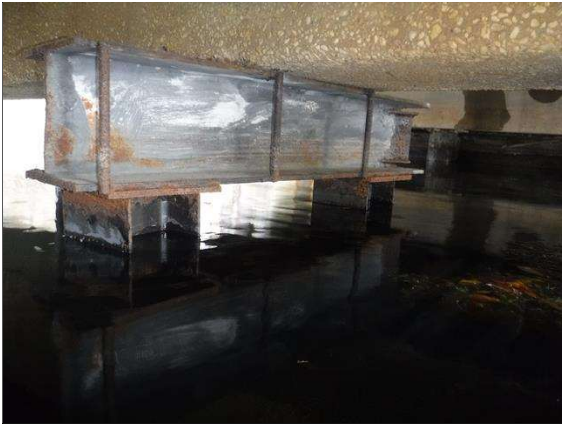
PILE 3 AT BENT 2 TEMPORARY SHORING, PILE 3 AT BENT 1 SIMILAR
