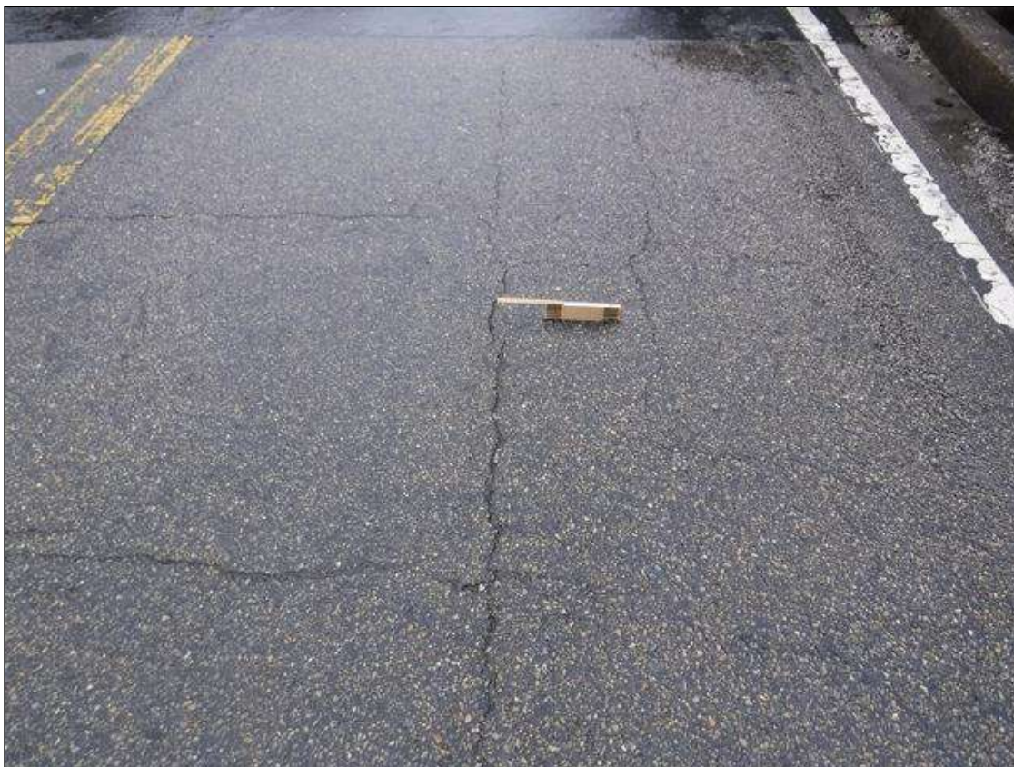
SCATTERED TRANSVERSE CRACKING / LONGITUDINAL CRACKING IN ASPHALT WEARING SURFACE UP TO AN .125" WIDE.
