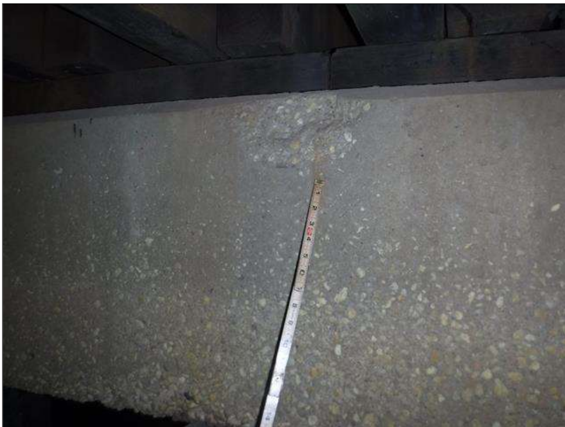
South face at top, above Steel Cross cap crutch, Spall no exposed steel (6" diameter x 1" deep.)
