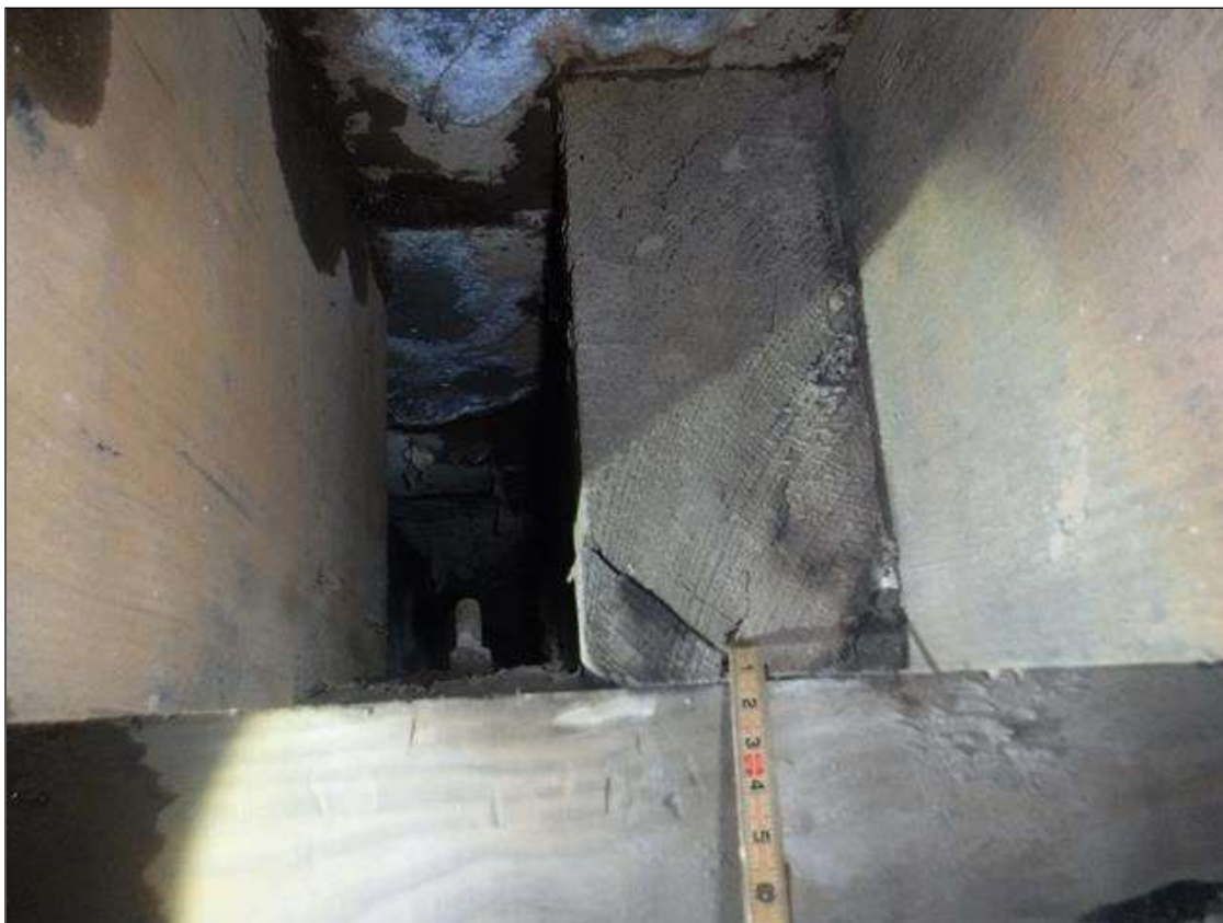
Span 1 Beam 10: UP TO 19" X 3" X 3" AREAS OF DELAMINATION IN BOTTOM CORNERS OF JOIST AT BENT 1
