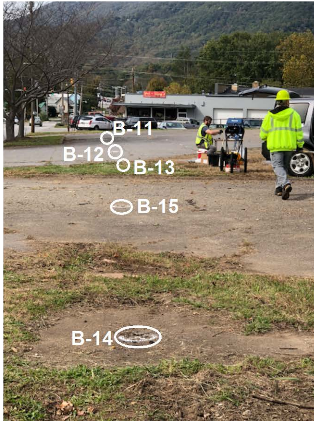
Describing and sampling Geoprobe cores. Driveway of former gas station is in the distance.
