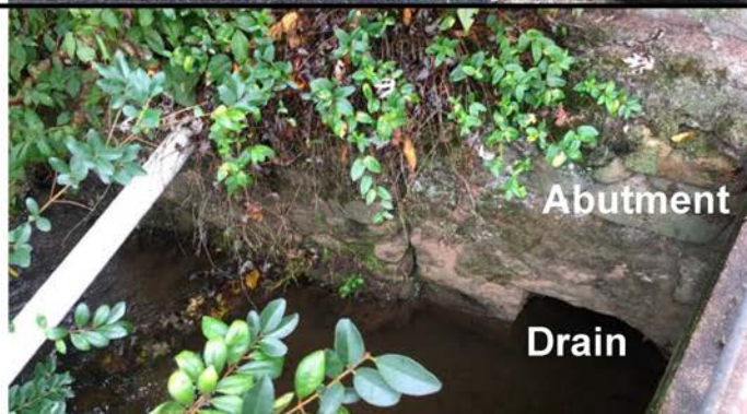
3. Stream at bridge abutment showing storm water drain (lower right) and PVC utility line that extend onto the property. Bridge abutment forms the northwest footing of the storage shed.
