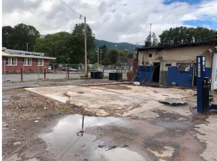
2. Building footing and remaining half of building at Parcel #008. Former restaurant building visible in background.
