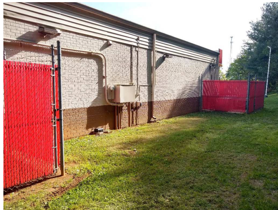
C. Photograph of rear of the gas station building with fenced-in air conditioning systems, looking southwest.
