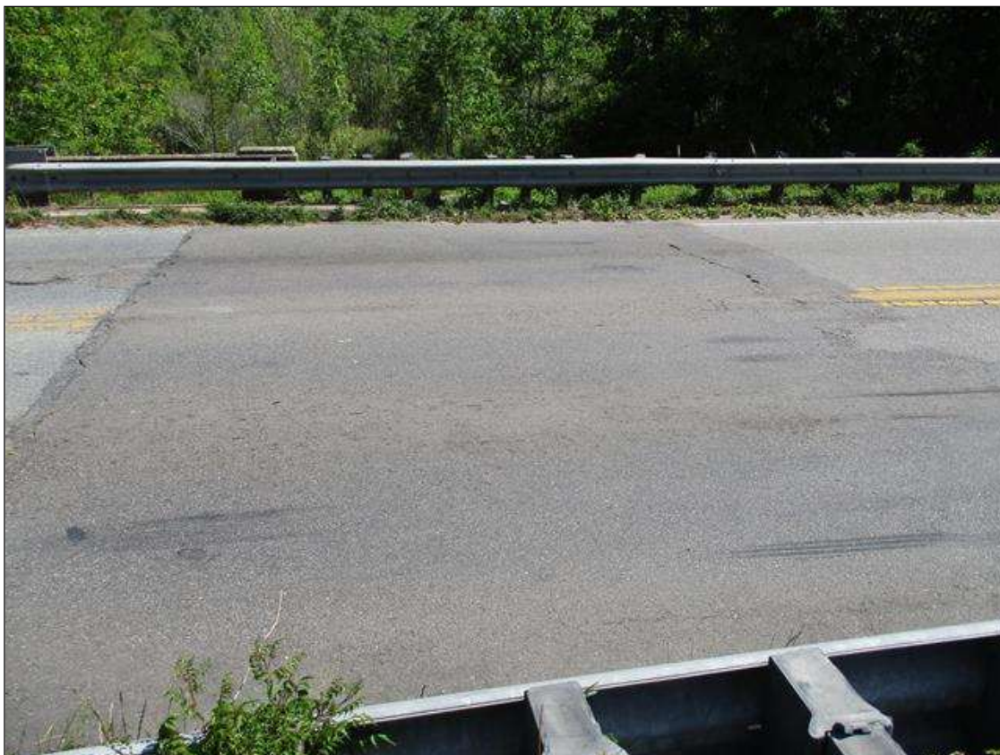
ASPHALT WEARING SURFACE SETTLED @ SOUTH END UP TO ( .5" TO 1" )
