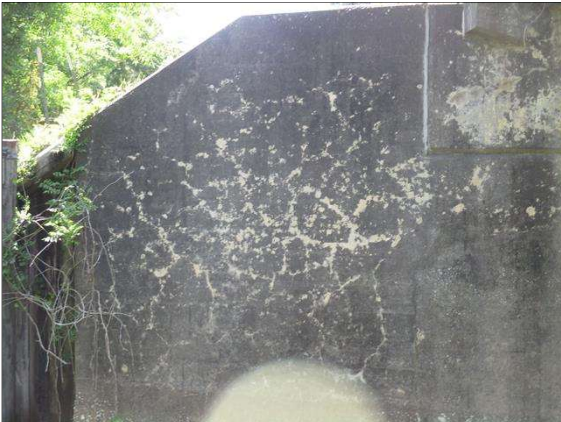
MAP CRACKING ( .020" WIDE ) WITH EFFLORESCENCE IN WEST AND EAST ENDS OF SOUTH AND NORTH ABUTMENTS ( EAST END OF SOUTH ABUTMENT SHOWN )
