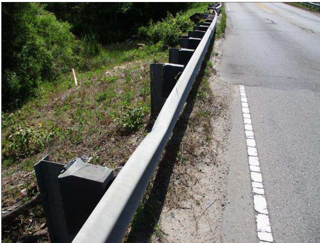
NORTHEAST APPROACH RAIL DAMAGED ( 25' LONG ) 75' FROM END BENT 2 ( PRIORITY ACTION REQUEST SUBMITTED )
