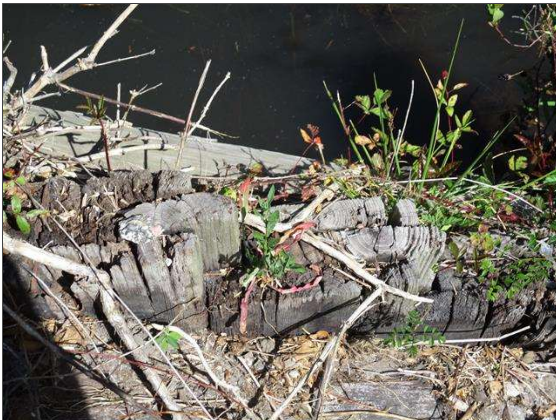
DECAY IN TOP PORTION OF VERTICAL WING WALL BOARDS ( 4" HIGH ) ( SOUTHEAST CORNER SHOWN )
