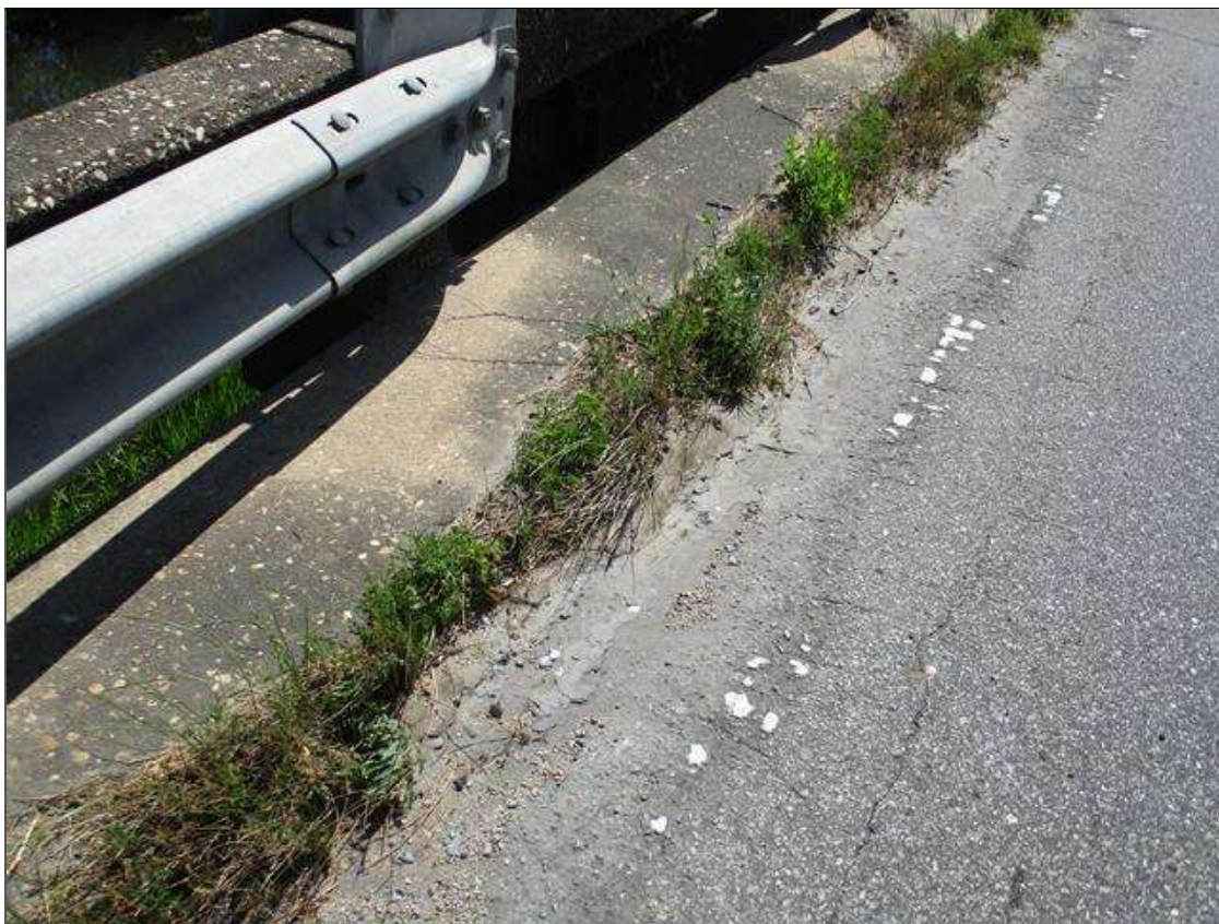
GROWTH AND DEBRIS ALONG WEST AND EAST RAILS BLOCKING DRAINS
