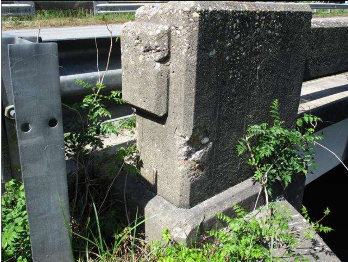
Span 1 Right Rail: SPALLED AREA ( 3" LONG X 5" WIDE X 5" HIGH ) NO EXPOSED REBAR IN POST # 1 EXTERIOR SIDE AT LOWER PORTION
