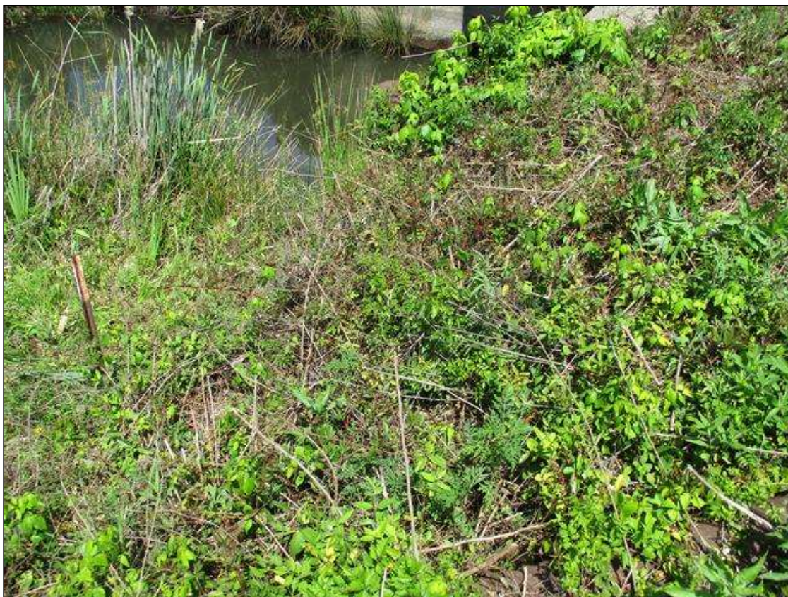
SINK HOLE ( 2' DIAMETER 1' DEEP ) BEHIND SOUTHWEST WING WALL
