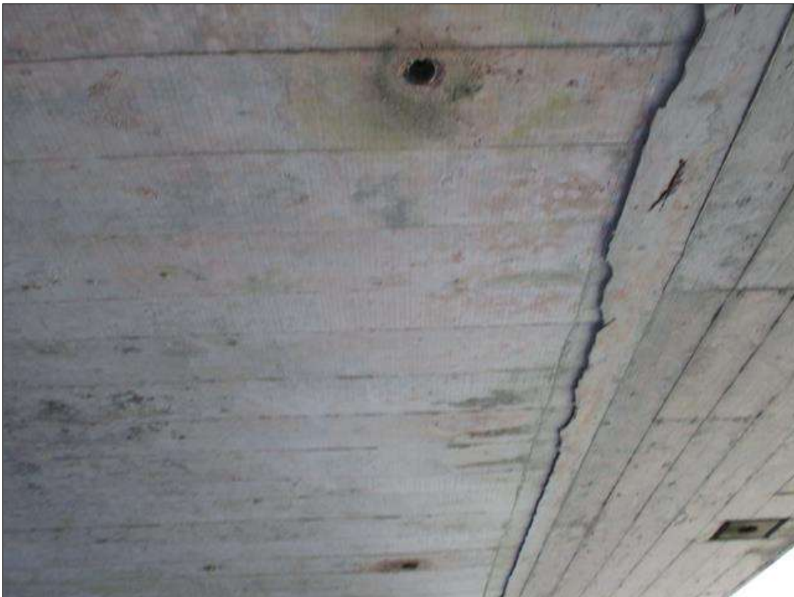
Span 1 Deck: 2 ( 2" ) SPALLED AREAS IN UNDERSIDE ( 6' FROM EAST SIDE )
