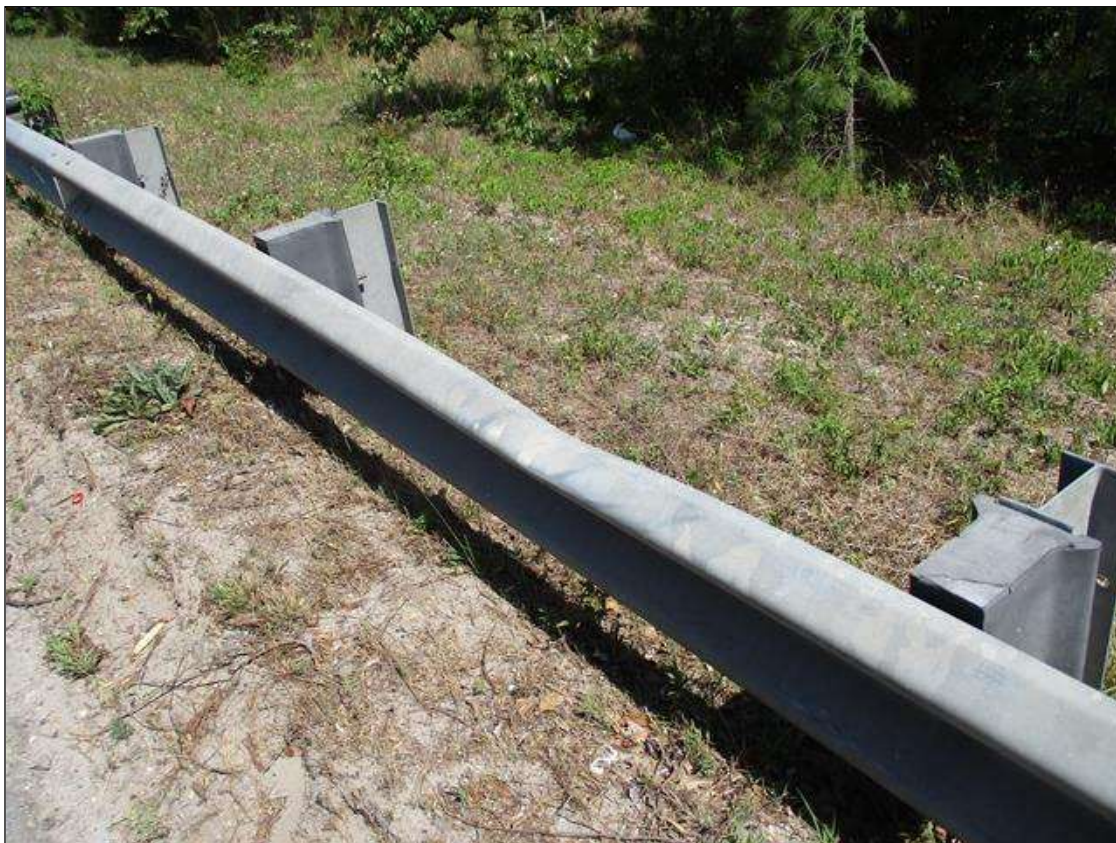
NORTHEAST APPROACH RAIL DAMAGED ( 25' LONG ) 40' FROM END BENT 2 ( PRIORITY ACTION REQUEST SUBMITTED )
