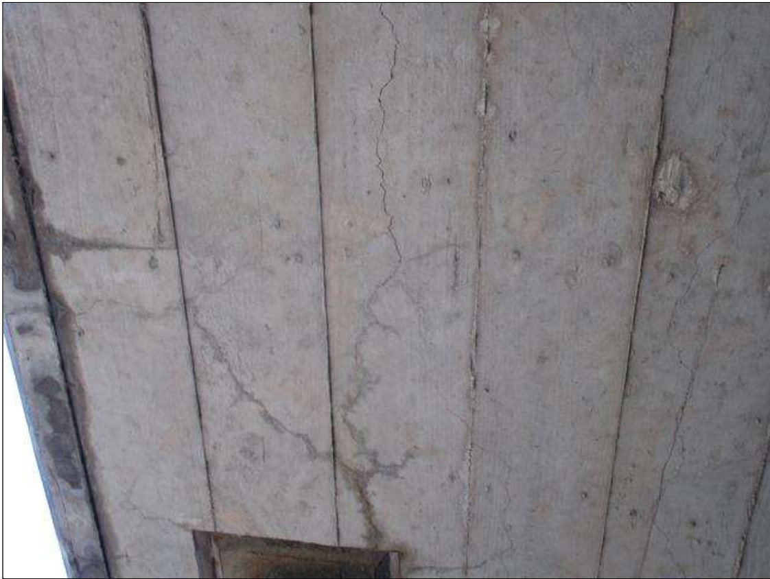
SCATTERED LONGITUDINAL CRACKING / MAP CRACKING ALONG UNDERSIDE OF DECK
