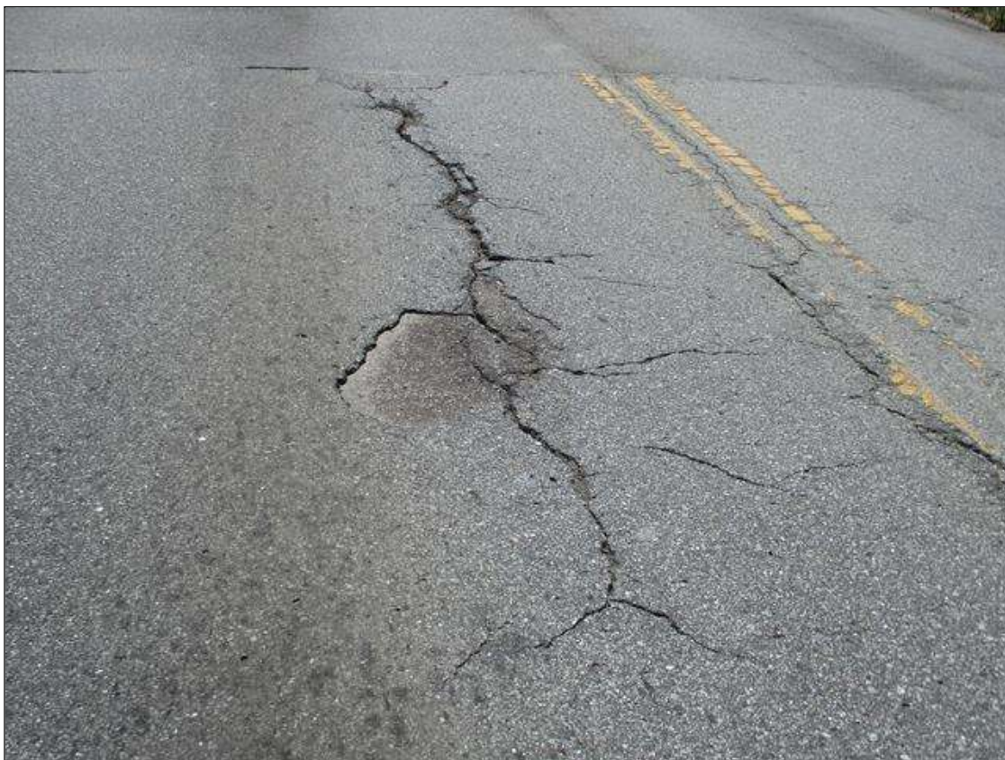
Wearing Surface: LONGIDUTINAL CRACKING (1" WIDE ) IN RIGHT LANE
