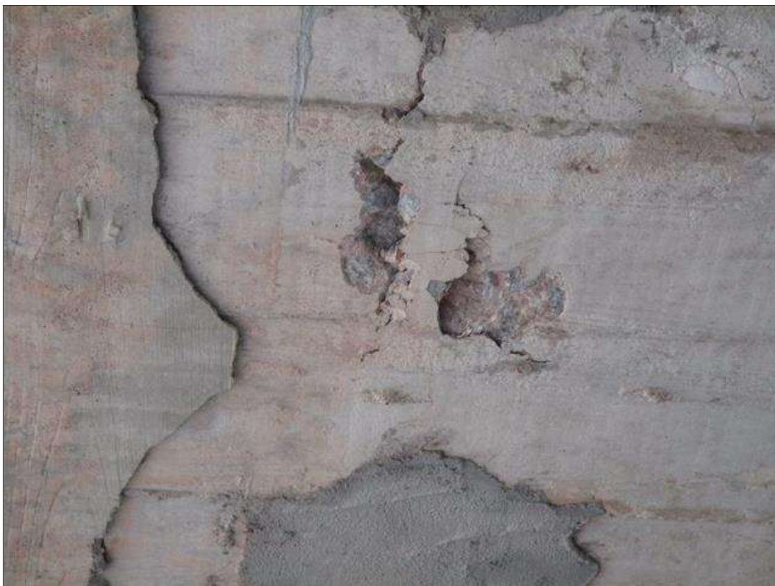
Span 1 Deck: SHALLOW SPALL/DELAMINATION ( 6" DIAMETER ) TO UNDERSIDE AT NORTH END WEST SIDE BETWEEN SOUND PATCHES
