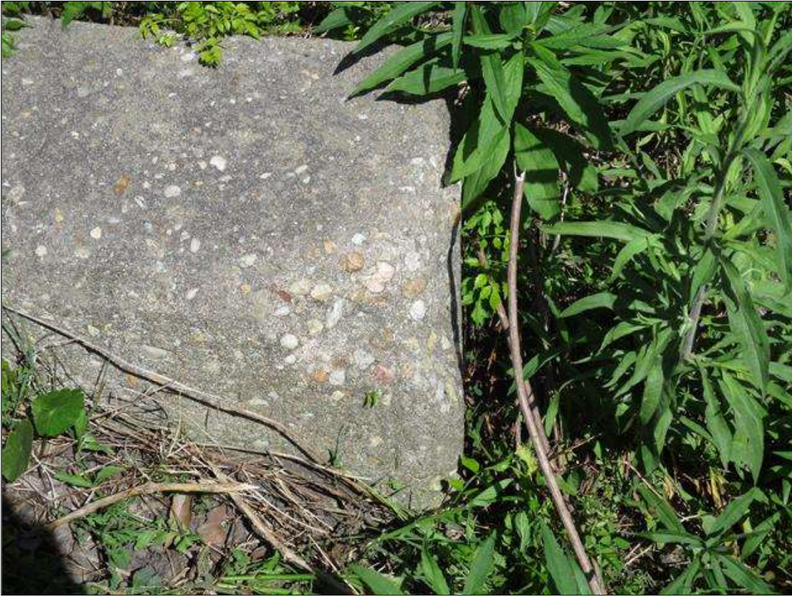
SPALL AREA ( 6" LONG X 4" WIDE X 4 " HIGH ) IN EAST CURB AT SOUTH END WITH NO EXPOSED REBAR
