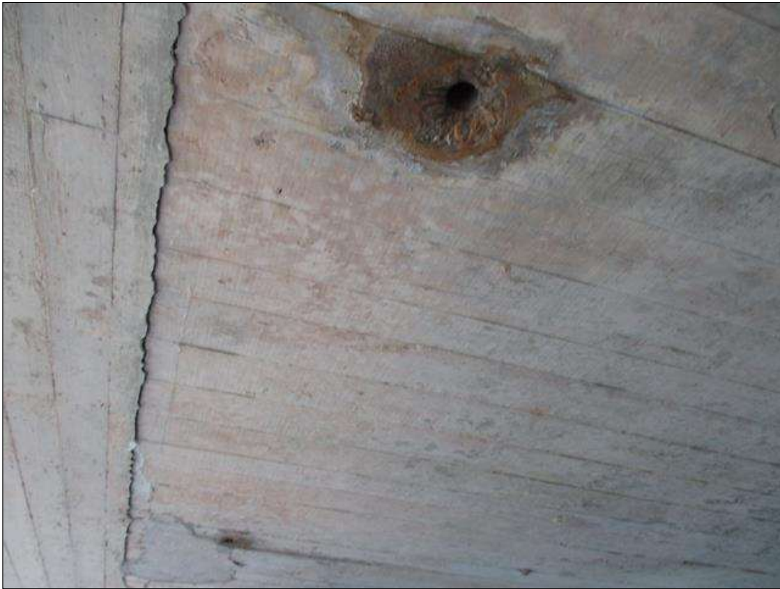
Span 1 Deck: 2 ( 2" ) SPALLED AREAS IN UNDERSIDE ( 6' FROM WEST SIDE )
