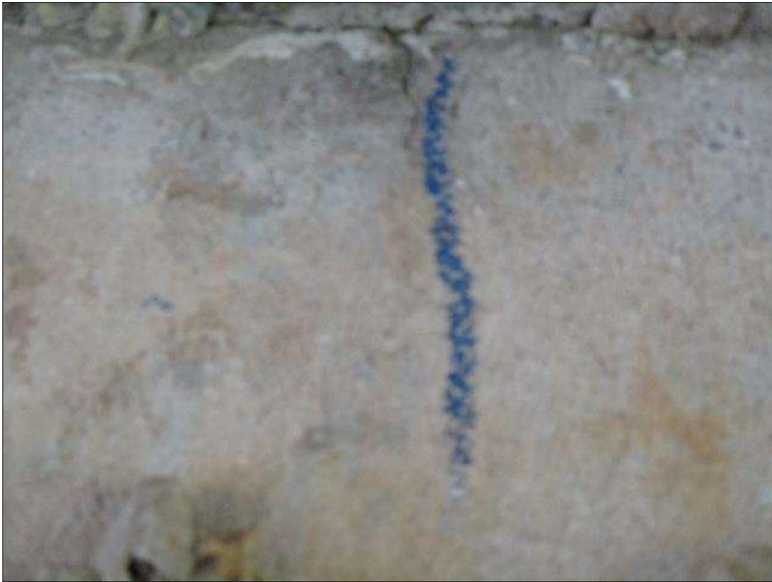
End Bent 2 Abutment: HAIRLINE VERTICAL CRACKING
