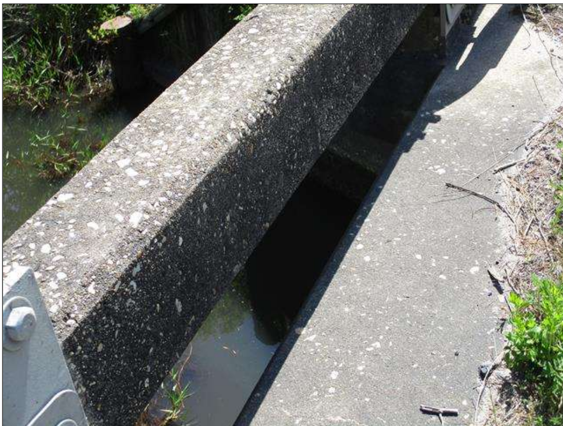
MODERATE WEAR WITH EXPOSED AGGREGATE THROUGHOUT WEST AND EAST RAILS
