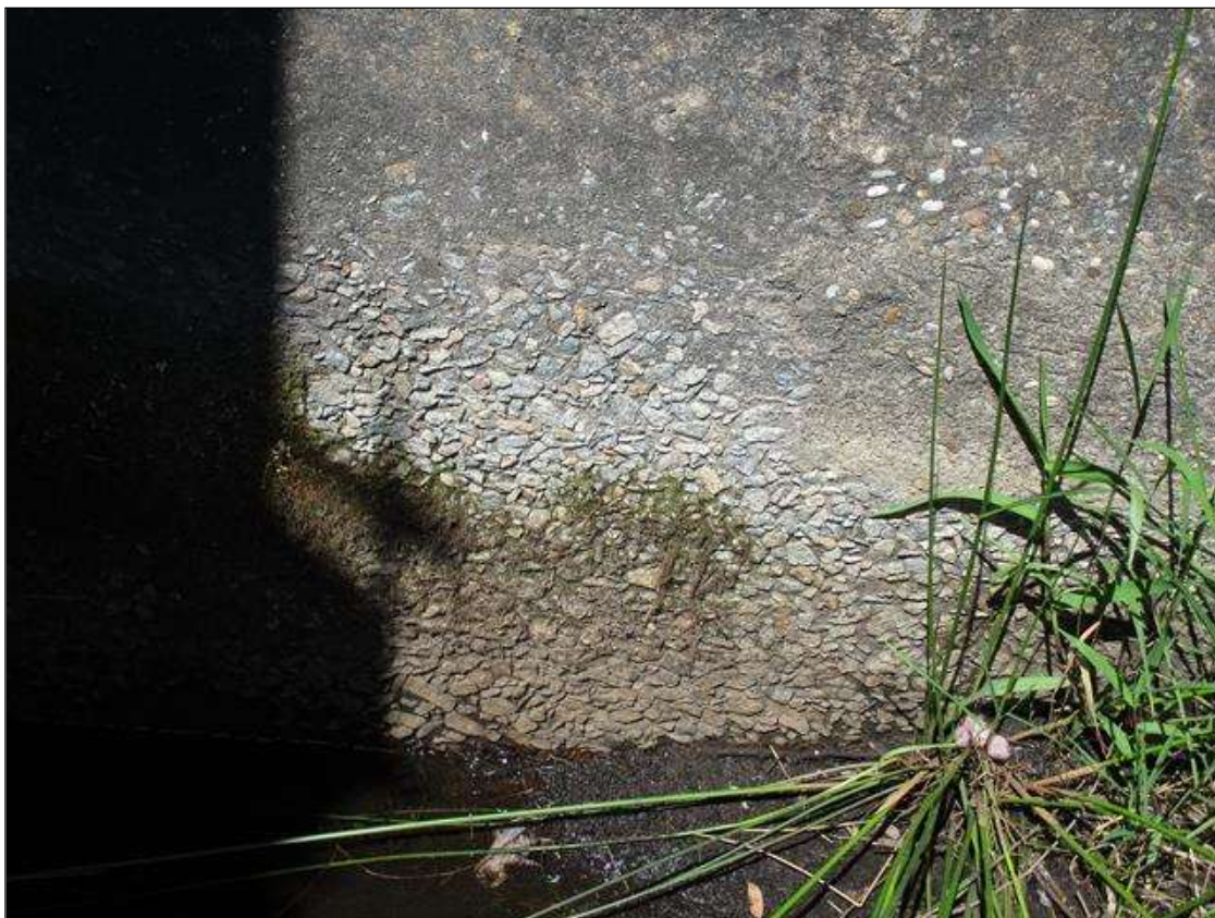
End Bent 1 Abutment: LOWER PORTION OF ABUTMENTS WORN WITH EXPOSED AGGREGATE
