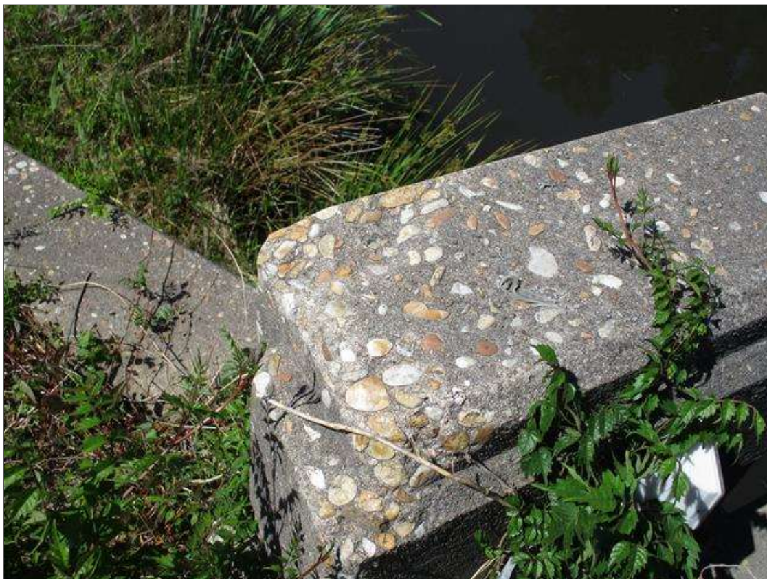
Span 1 Left Bridge Rail: SPALLED AREA (8" LONG X 5" WIDE X 1" HIGH) IN THE TOP PORTION OF THE SOUTHEAST RAIL POST
