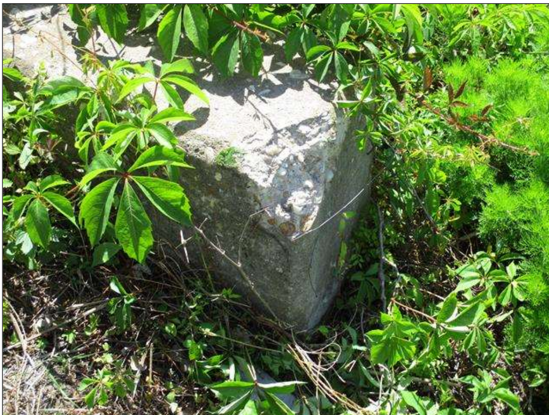
SPALL AREA ( 4" LONG X 6" WIDE X 4" HIGH ) IN WEST CURB AT NORTH END WITH NO EXPOSED REBAR
