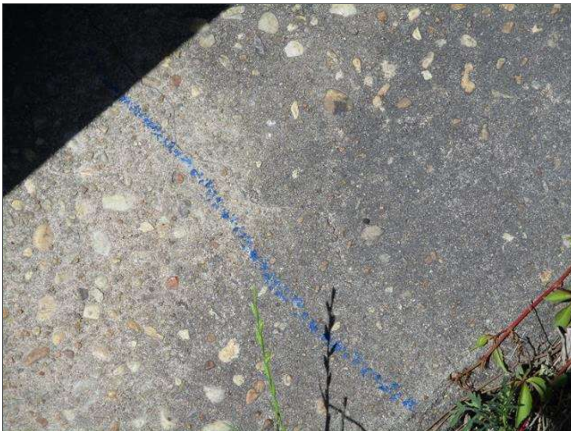
Span 1 Left Bridge Rail: SCATTERED CRACKING IN CURBS (.062" WIDE)
