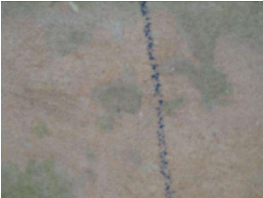
End Bent 1 Abutment: HAIRLINE VERTICAL CRACKING
