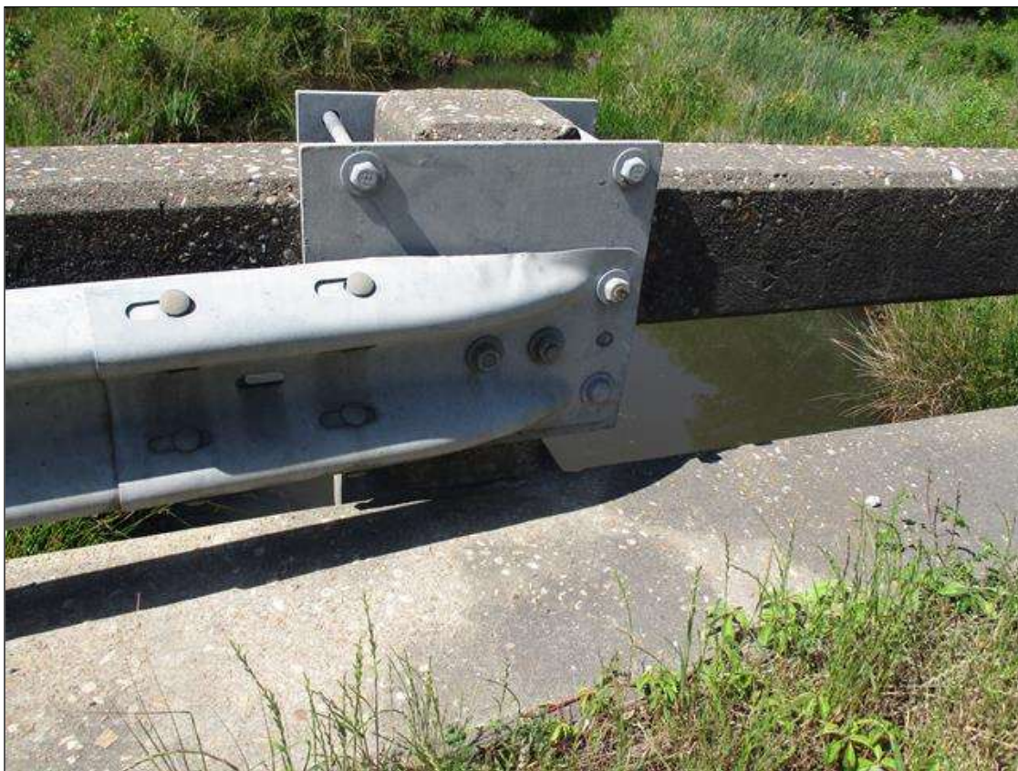
SIMILAR GUARDRAIL CONNECTION ( SOUTHWEST SHOWN )
