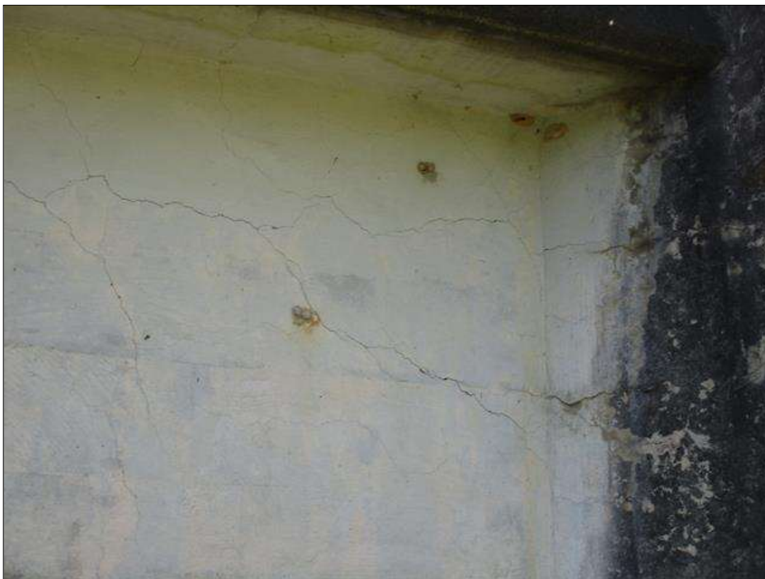
Span 1 Deck: MAP CRACKING ALONG EXTERIOR SIDES OF DECK UP TO .025" WIDE
