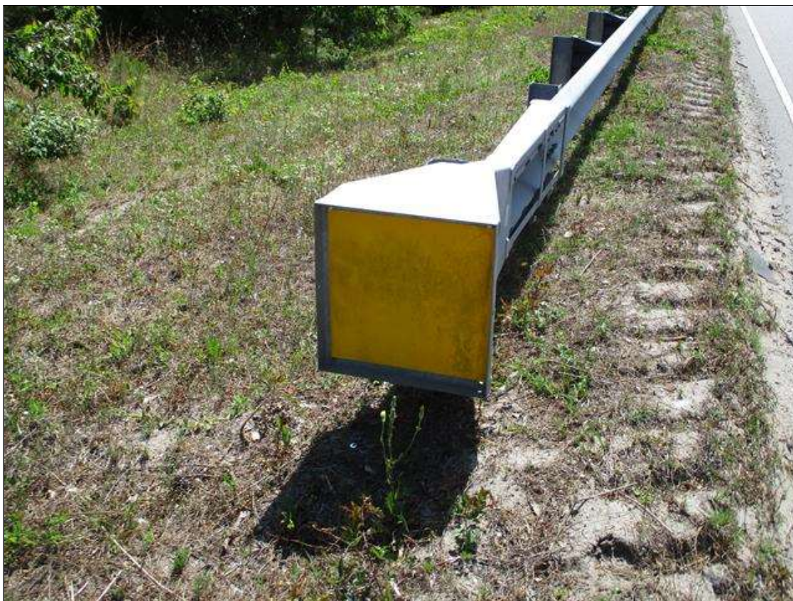
NORTHEAST GUARDRAIL END TERMINAL
