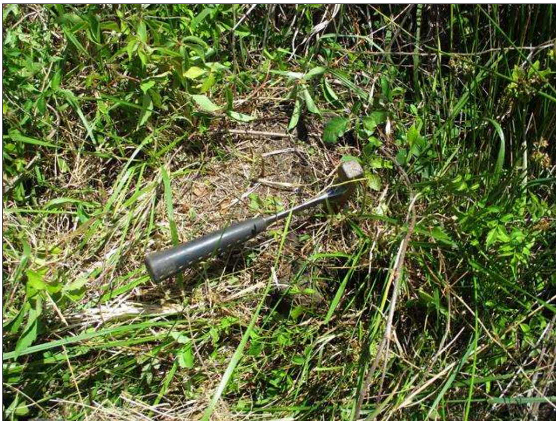
NORTHWEST WING PILE #2 DECAYED ( 1/2 CIRCUMFERENCE X 6" HIGH )
