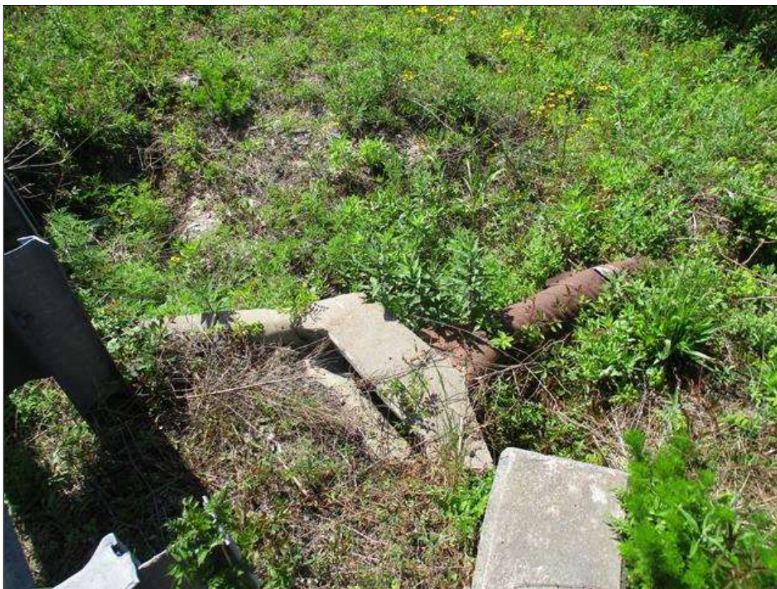
EROSION ( 8' LONG X 10' WIDE X 1.5' DEEP ) @ SOUTHWEST APPROACH CORNER DRAIN
