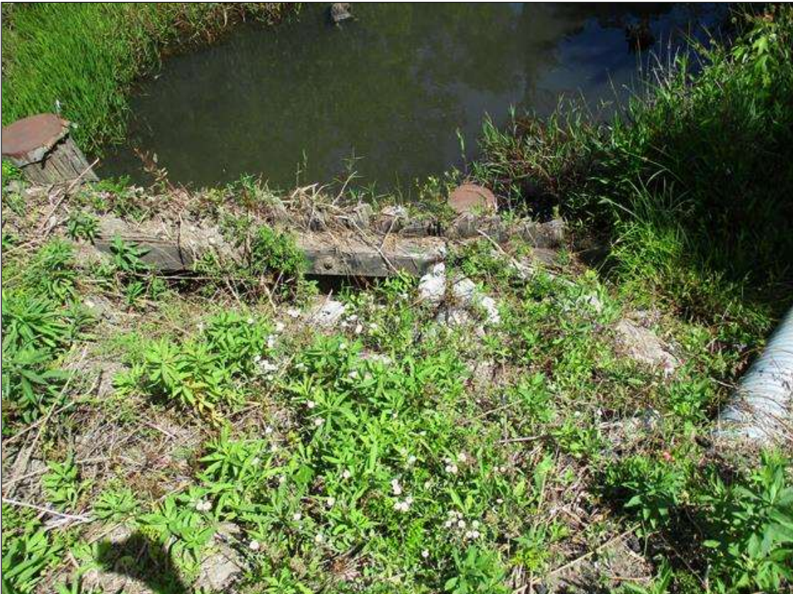
EROSION ( 8" LONG X 10' WIDE 1' TO 1.5' DEEP ) AT SOUTHEAST CORNER WING WALL
