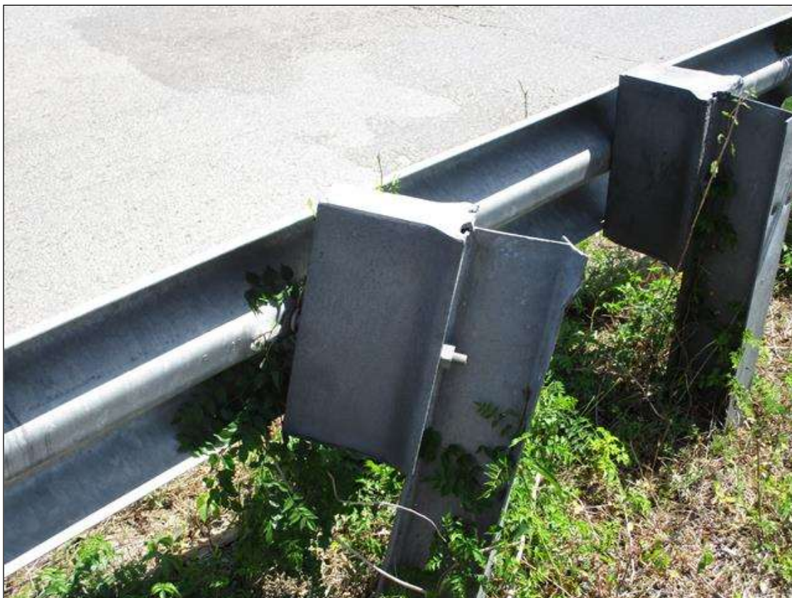
NORTHWEST GUARDRAIL POST DAMAGED ( 25' FROM END BENT 2 ) ( PRIORITY ACTION REQUEST SUBMITTED )
