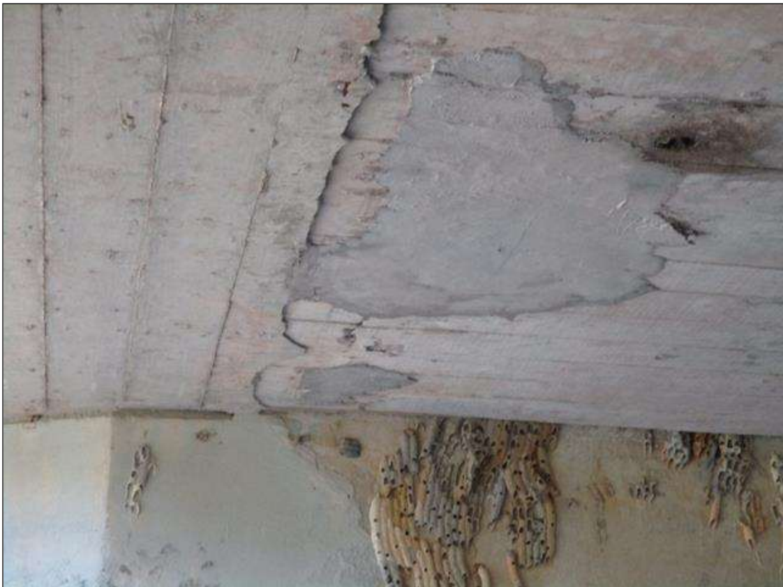
2 SOUND PATCHES TO UNDERSIDE AT NORTH END WEST SIDE
