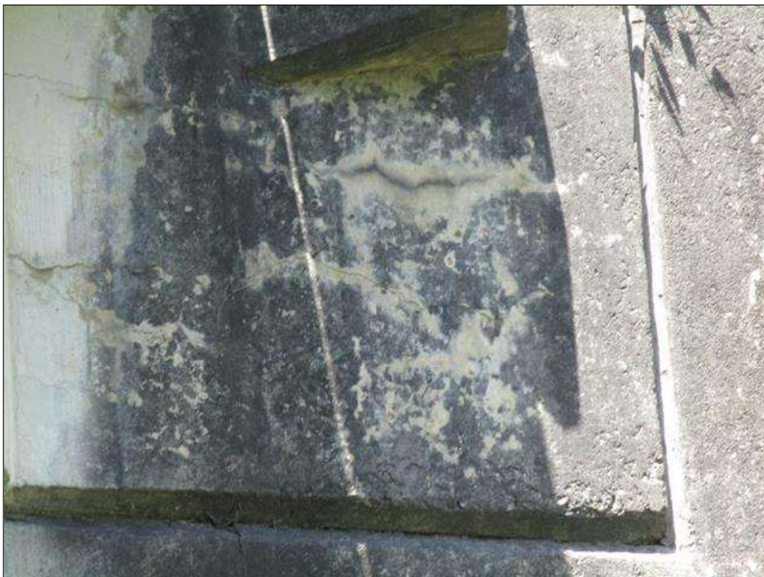
HORIZONTAL CRACKING (HAIRLINE TO 1/32IN) AND MAP CRACKING AT WEST AND EAST ENDS OF SOUTH AND NORTH ABUTMENTS ( NORTH ABUTMENT EAST END SHOWN )
