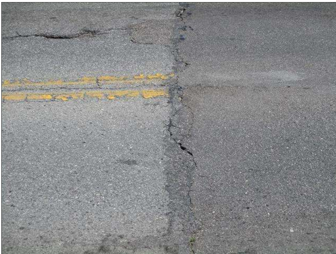
TRANSVERSE CRACKING IN ASPHALT WEARING SURFACE (.250" WIDE) OVER END BENT 1
