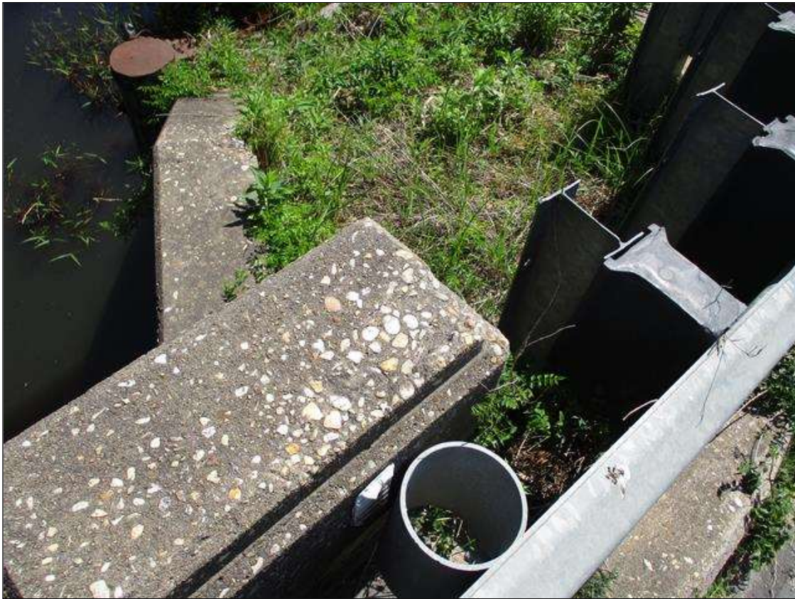
Span 1 Right Bridge Rail: SPALLED AREA (6" LONG X 3" WIDE X 1" HIGH) THE TOP PORTION OF THE SOUTHWEST RAIL POST.
