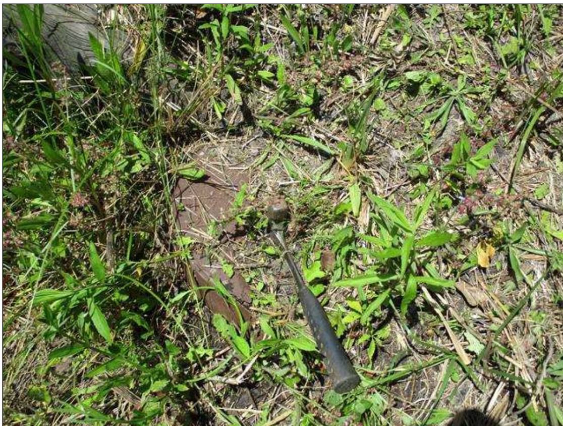
NORTHEAST WING PILE #2 DECAYED ( 1/2 CIRCUMFERENCE X 6" HIGH )
