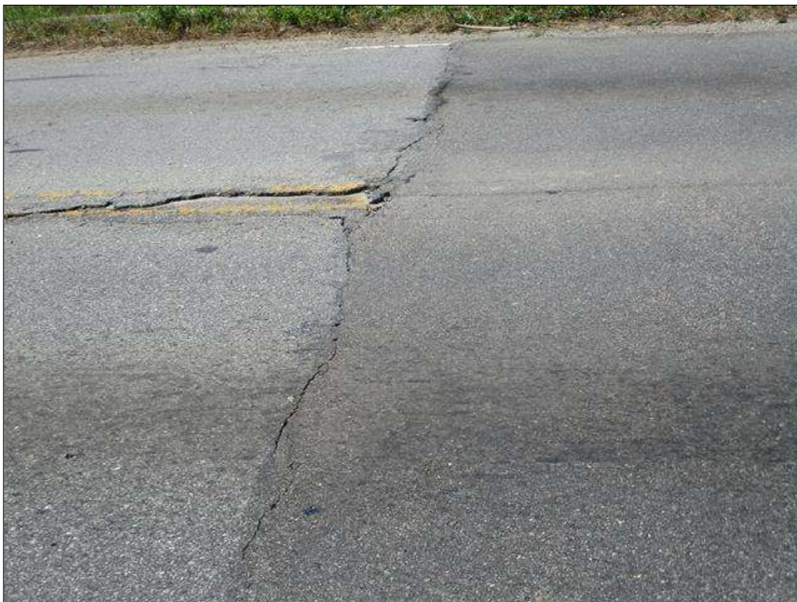
TRANSVERSE CRACKING IN ASPHALT WEARING SURFACE (.250" WIDE) OVER END BENT 2
