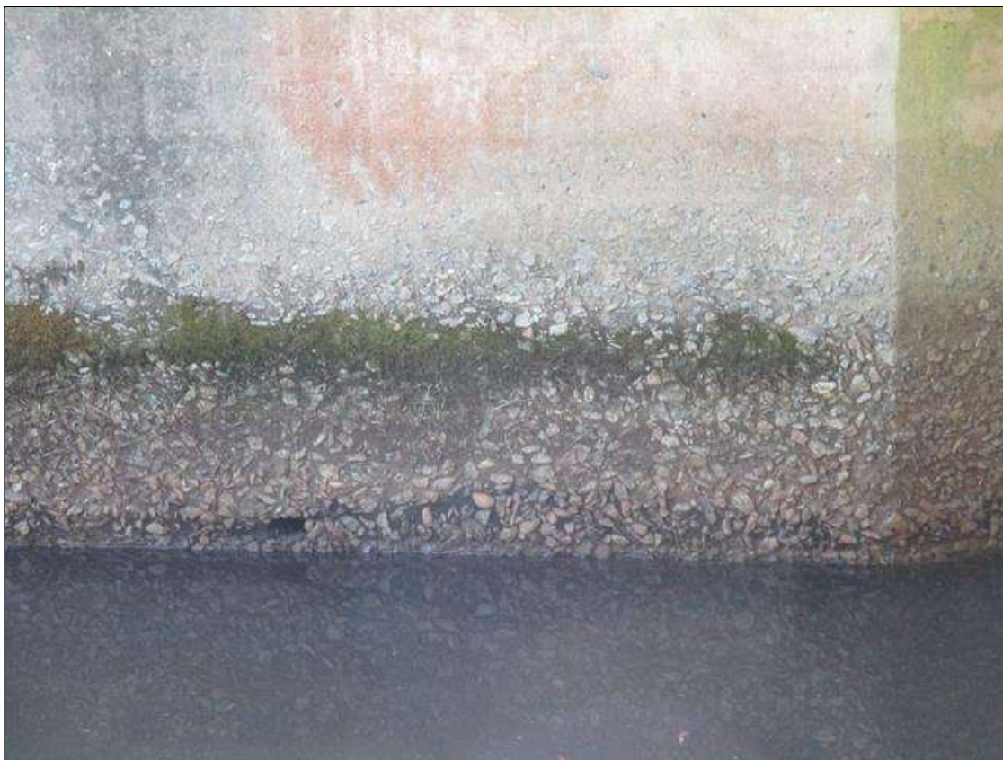
End Bent 2 Abutment: LOWER PORTION OF ABUTMENTS WORN WITH EXPOSED AGGREGATE
