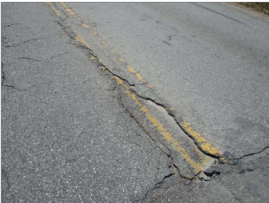
Span 1 Wearing Surface: SPALL (6' LONG X 1' WIDE X .5" DEEP ) AT CENTERLINE AT NORTH END.
