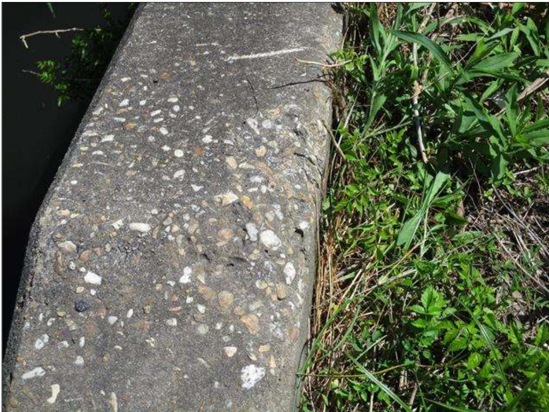
End Bent 1 Abutment: SPALLED AREA ( 1' LONG X 4" WIDE X 1" HIGH ) WITH NO EXPOSED REBAR AT EAST END TOP PORTION
