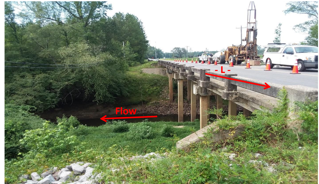
Photograph No. 4: View from East Side of bridge looking South, drilling B1-A
