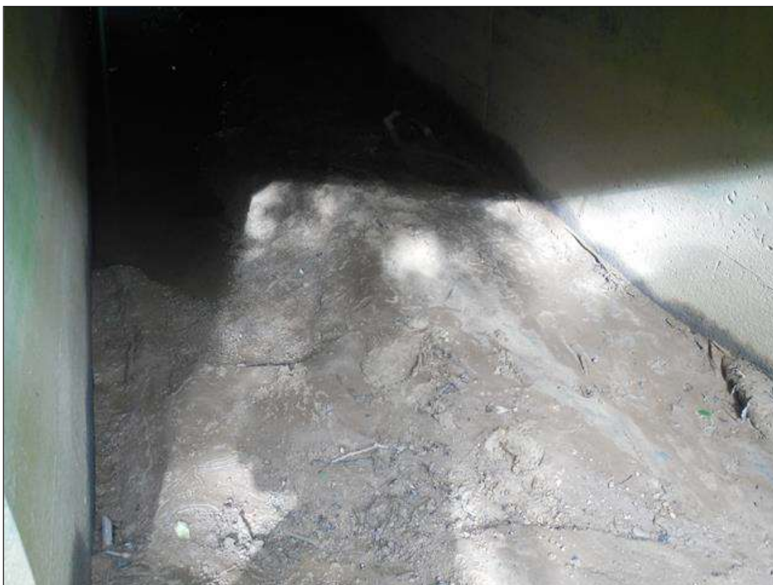
BARREL 2 HAS UP TO 3FT OF PARTIAL SILT ALONG LENGTH.
