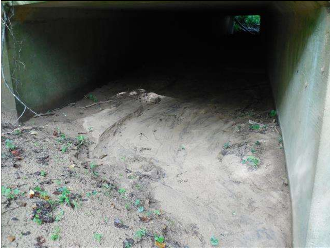
BARREL 1 HAS UP TO 5FT OF SILT ALONG LENGTH.
