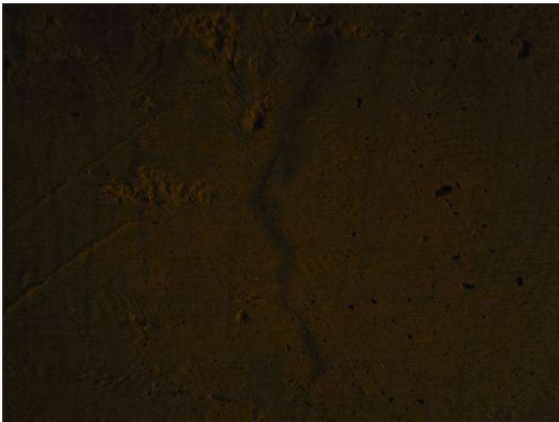
Span 3 Culvert Section 1: H/L VERTICAL CRACKING
