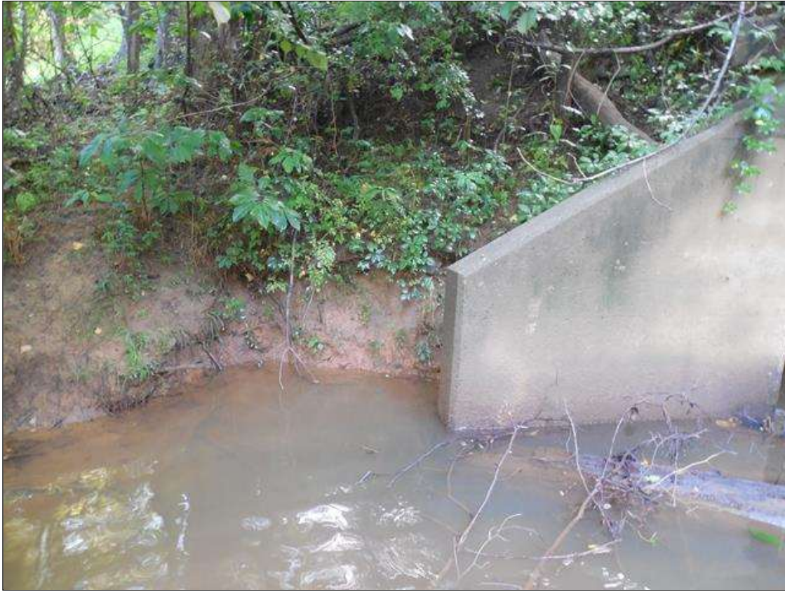
NORTHWEST WINGWALL IS WASHING BEHIND IT IN A 5FT X 5FT AREA .
