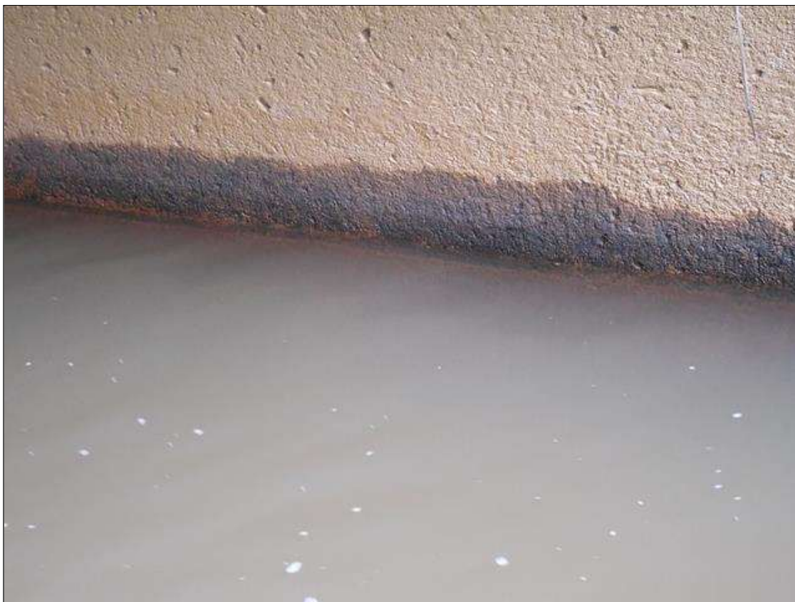
Span 3 Culvert Section 1: 1/8" PITTING ALONG THE WATERLINE
