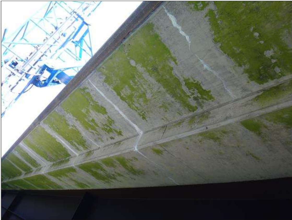
Span 2 Deck: underside East overhang scattered throughout, multiple transverse cracks [full width x hairline] with efflorescence, West overhang similar
