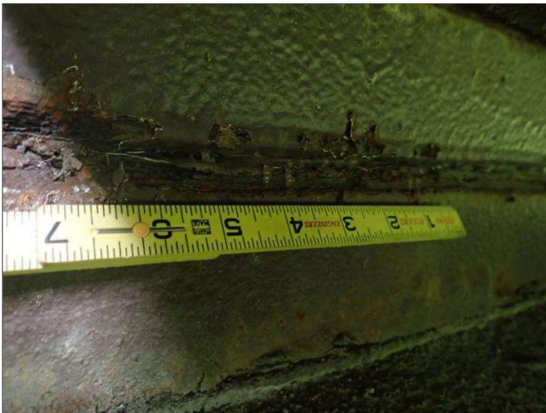
Span 1 Beam 2 Near Bearing: active corrosion with section loss [loss up to 1/8in] with pack rust [1/2in]
