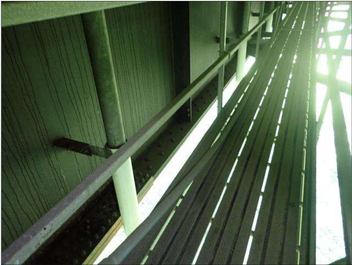
Utilities: span 2 beam 1 between floor beam 3 and 4, attached utility broken and detached
