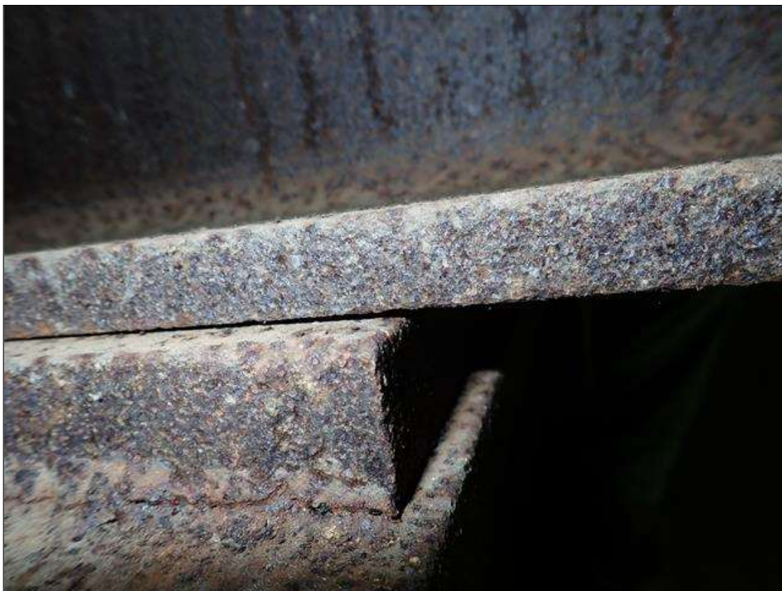
Span 2 Stringer 2: [PAR] at floor beam 33, missing anchor bolts on East face and two cracked tack welds [full length]
