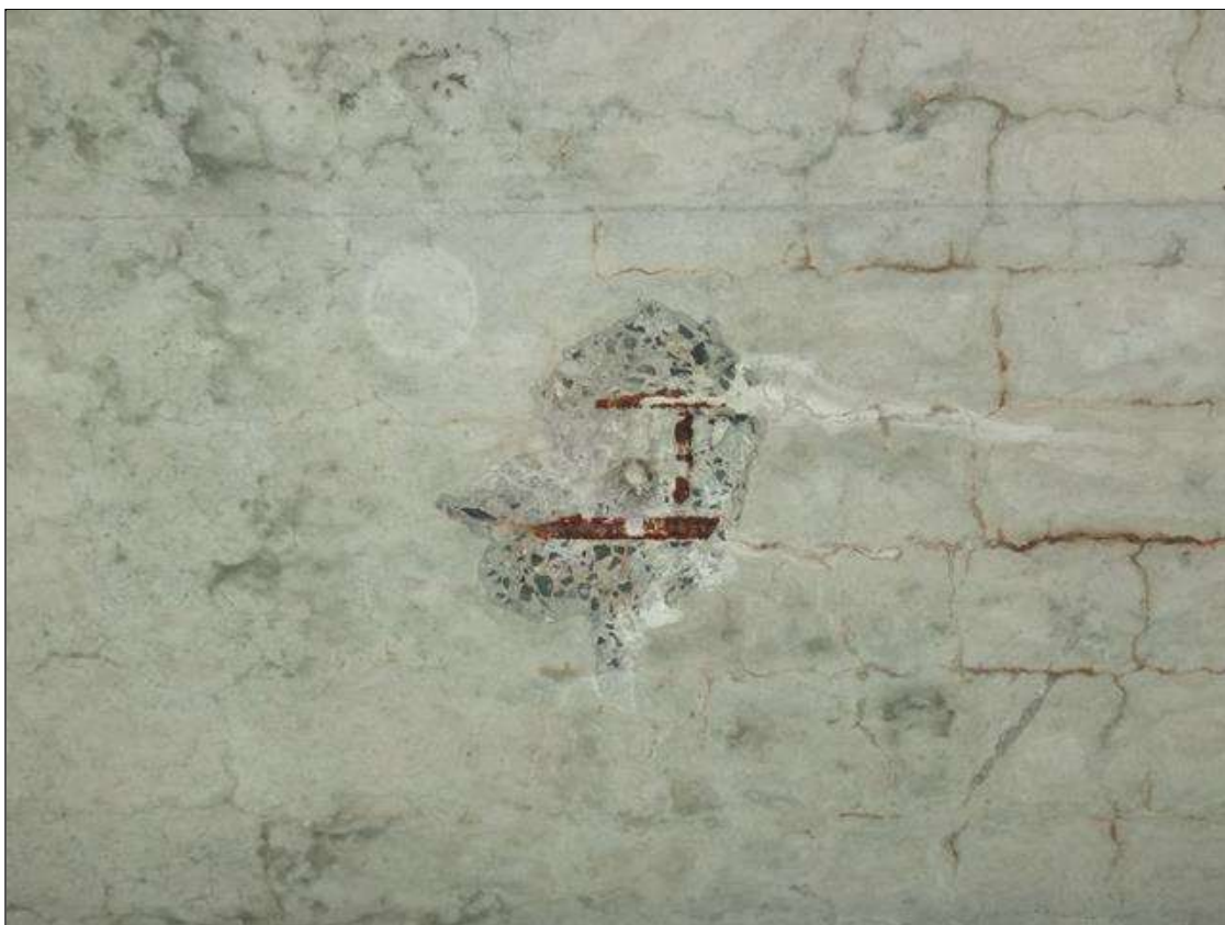
Span 4 Deck: [PAR] underside of deck at far end, spall [12in x 12in x 3in deep] with exposed transverse and longitudinal rebar [loss < 1/16in]
