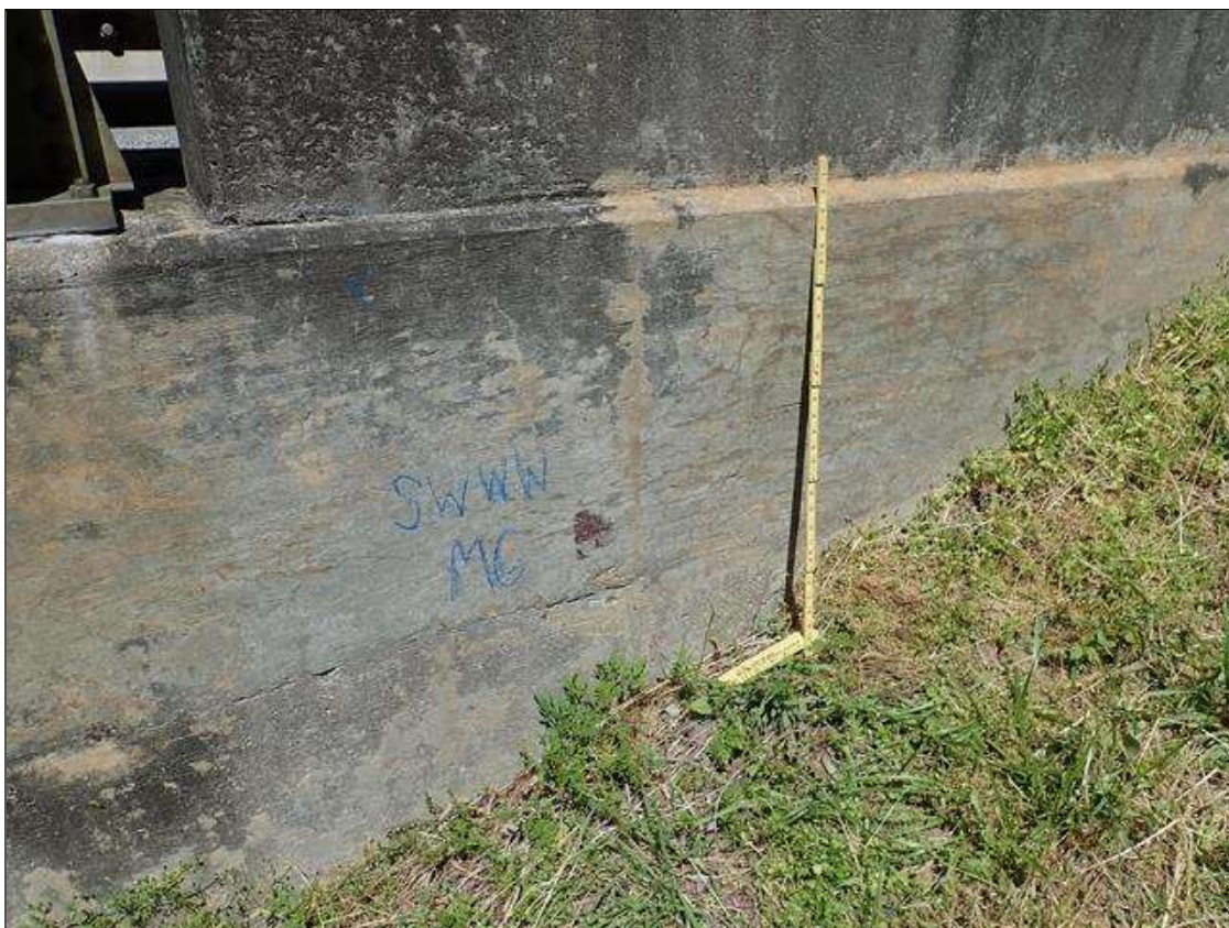
Southwest wingwall: left side at near end, hairline map cracking with efflorescence [8ft x 2ft]
