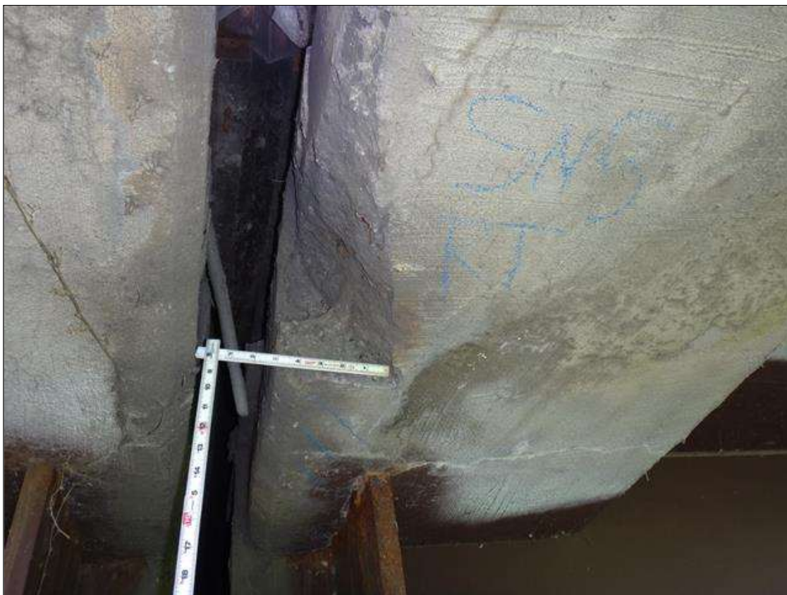
Span 5 Deck: underside East overhang at bent 4, spall [36in x 6in x 8in deep]
