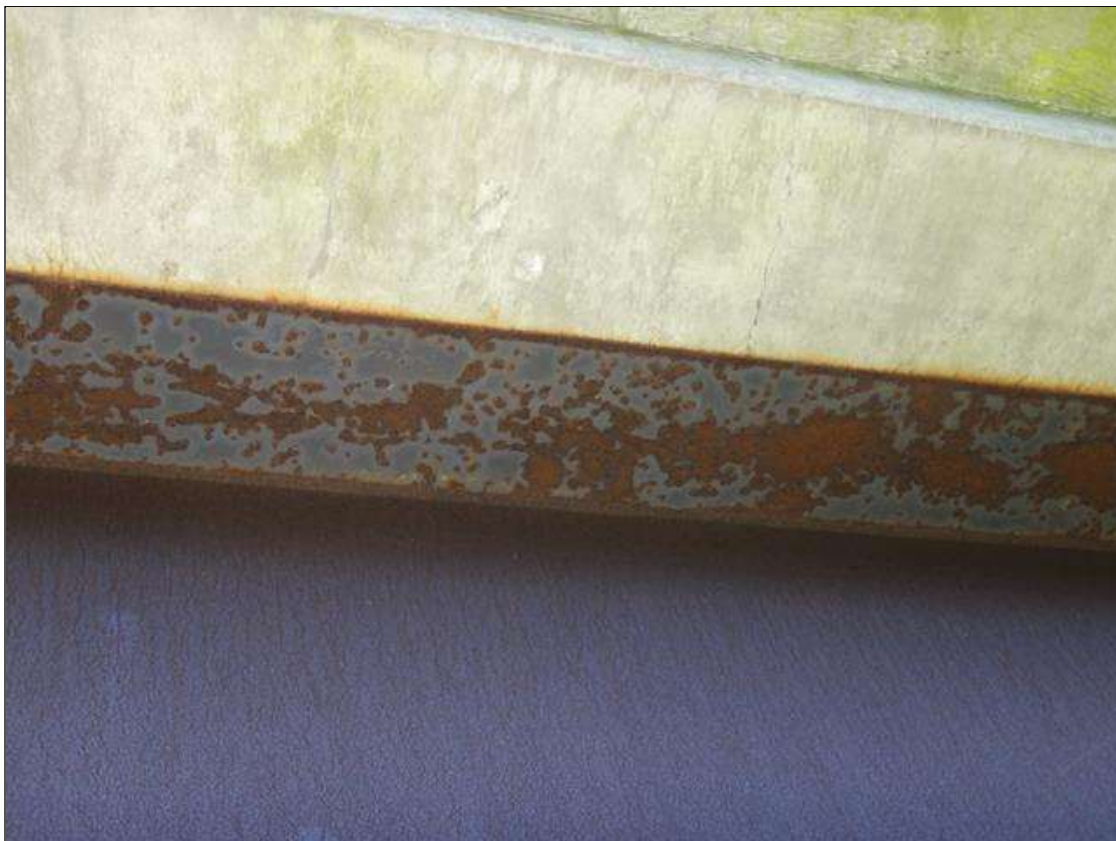
Span 2 Beam 1: underside of top flange over bent 3, underdeveloped patina with exposed steel
