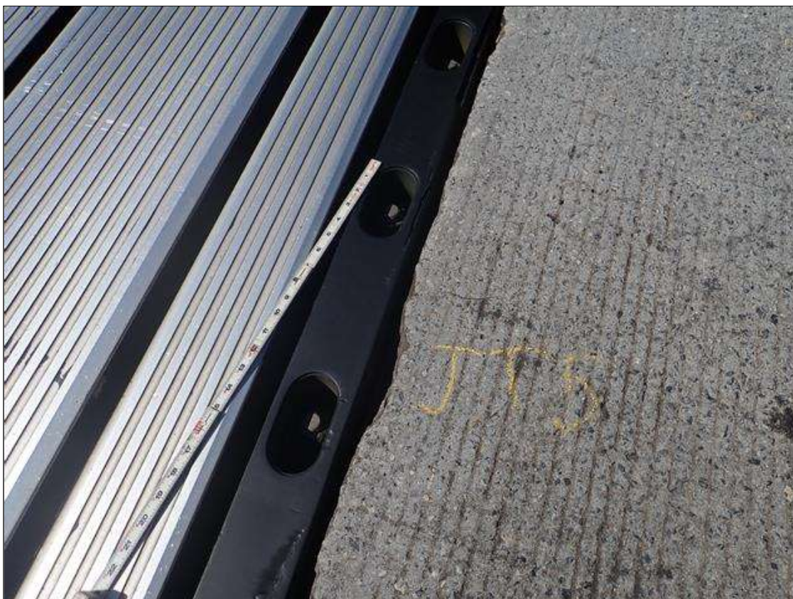
Expansion Joint 2 : at both sides of joint, missing plug covers [up to full length]
