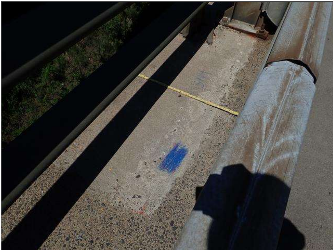
Span 4 Left Bridge Rail: curb at midspan, sound patch [8ft x 2.5in]
