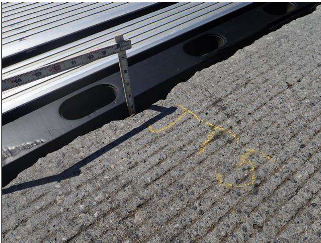
Expansion Joint 2 : along length of joint, missing joint sealant material [up to 28ft]
