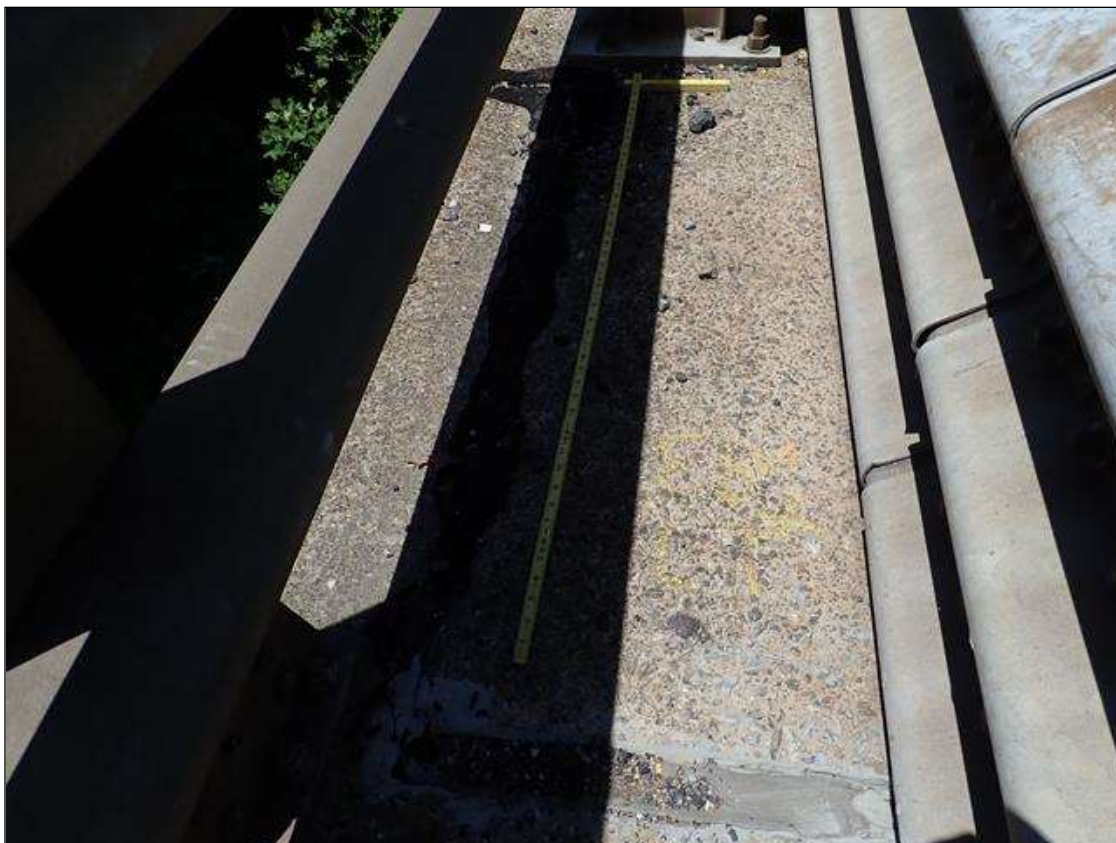
Span 1 Left Bridge Rail: over end bent along joint between wingwall and curb, loss of seal adhesion [up to 4ft] similar at all corners
