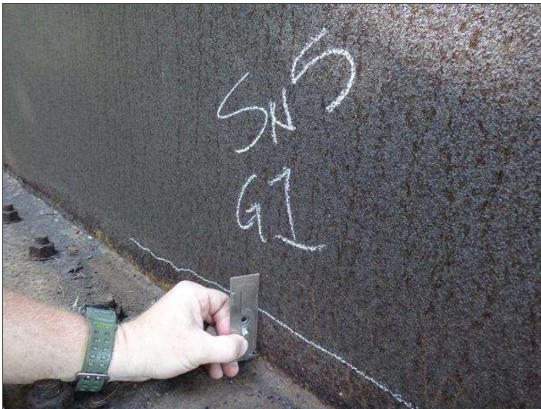
Span 1 Beam 2: lower web along length of exterior face, active corrosion with section loss [85ft x up to 2-1/2in x up to 3/32in deep]
