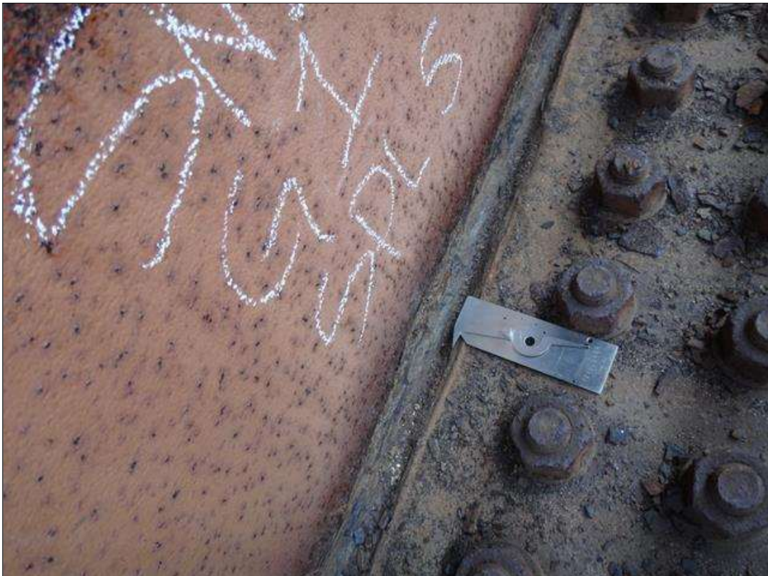
Span 2 Beam 1: [PAR] span 2, exterior and interior of lower web at splice 5, active corrosion with section loss [7ft x 2-1/2in - avg rem 7/16in] with areas of up to 1/4in loss [avg rem 3/8in]
