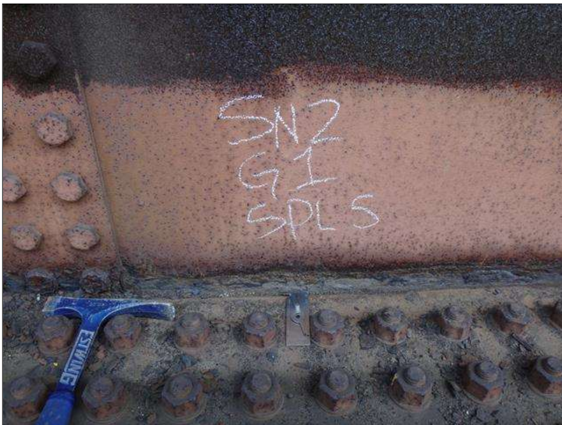
Span 2 Beam 1: [PAR] span 2, exterior and interior of lower web at splice 5, active corrosion with section loss [7ft x 2-1/2in - avg rem 7/16in] with areas of up to 1/4in loss [avg rem 3/8in]
