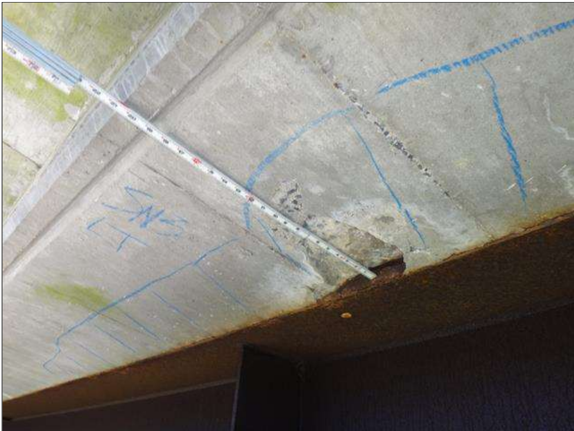
Span 3 Deck: underside left overhang at web stiffener 21, spall/delamination [7ft-10in x 13in x 1-1/4in deep] with pack rust between top flange and deck [1/4in]
