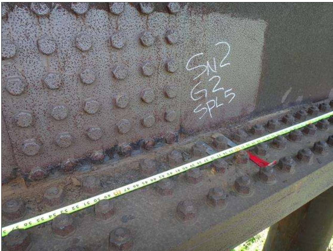
Span 2 Beam 2: [PAR] lower web exterior face at splice 5, active corrosion with section loss [7ft-10in x up to 2-1/2in - avg rem 15/32in]
