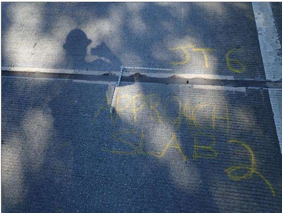
Expansion Joint 1 : at 5ft from East curb, hole in joint material [1-1/2in x 1/2in x 1-3/4in deep]
