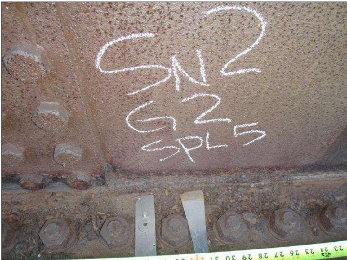
Span 2 Beam 2: [PAR] lower web exterior face at splice 5, active corrosion with section loss [7ft-10in x up to 2-1/2in - avg rem 15/32in]
