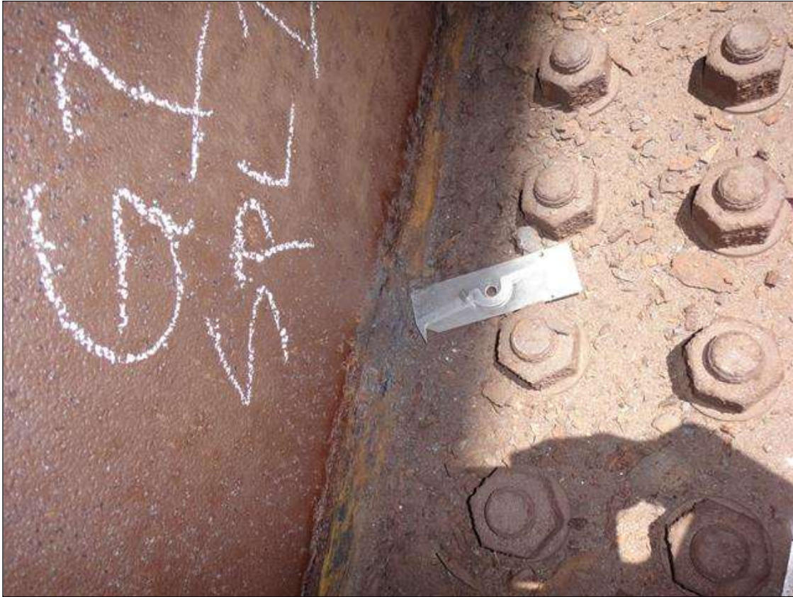
Span 2 Beam 1: span 3, lower web and splice plate both faces at splice plate 11, active corrosion with section loss, web [6.5ft x 3in - avg rem 1/2in] with areas of 3/16in loss [avg rem 3/8in]; plate [full width x 1-1/2in x 1/16in loss], and lower bolts [10% loss]
