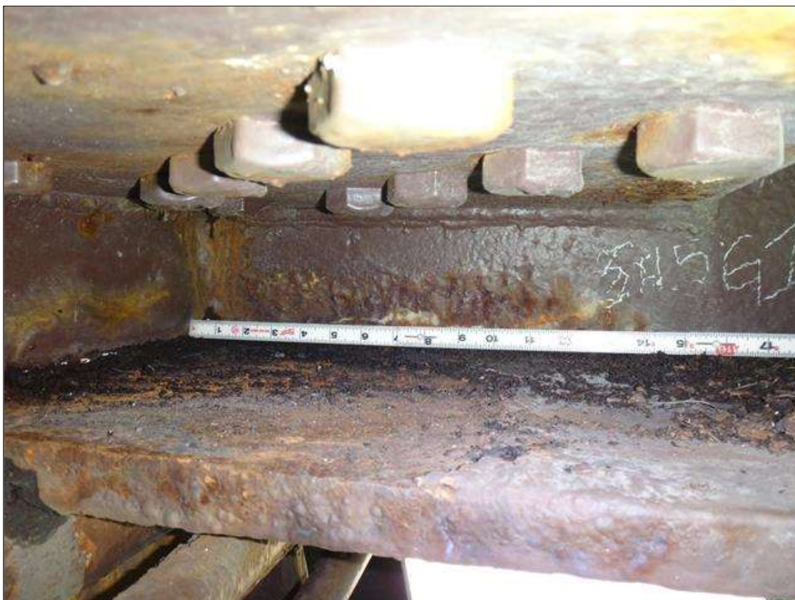
Span 1 Beam 2: [PAR] at bent 1, arrested metal loss, lower web [18in x 3in - avg rem 1/4in]; bottom flange [18in x 12in - avg rem 7/8in]
