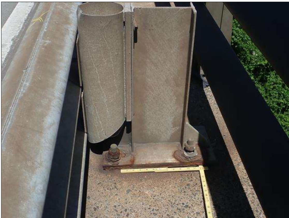
Span 1 Right Bridge Rail: along length of thrie beam at base of posts, active surface corrosion and some with pack rust
