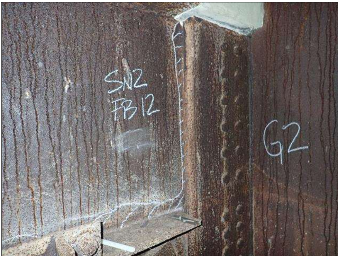
Span 2 Floor Beam 12: lower web South face next to girder 2, active corrosion with section loss [full height x up to 2in - avg rem 3/8in] with pack rust [up to 5/16in]
