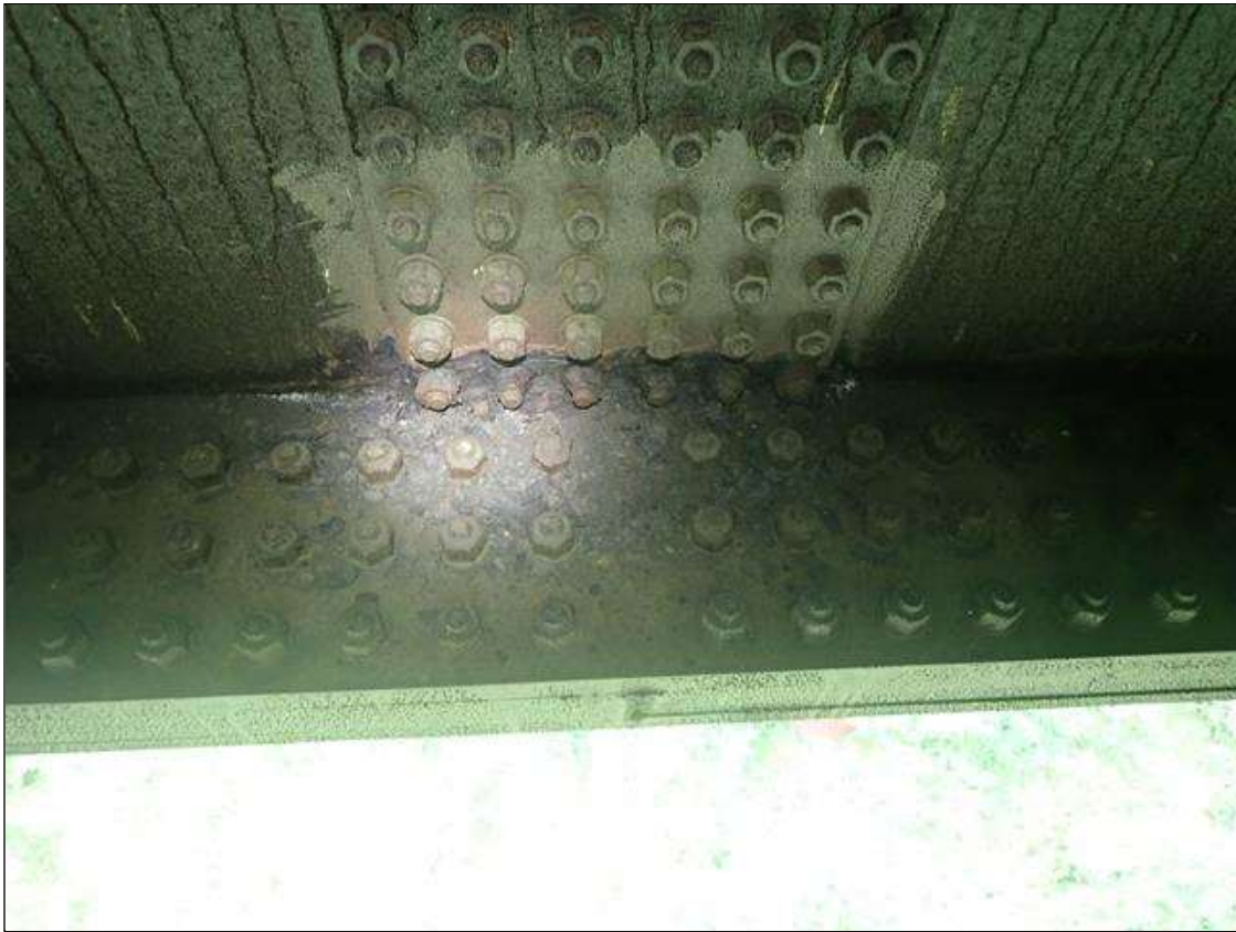
Span 2 Beam 1: span 3, lower web and splice plate both faces at splice plate 11, active corrosion with section loss, web [6.5ft x 3in - avg rem 1/2in] with areas of 3/16in loss [avg rem 3/8in]; plate [full width x 1-1/2in x 1/16in loss], and lower bolts [10% loss]
