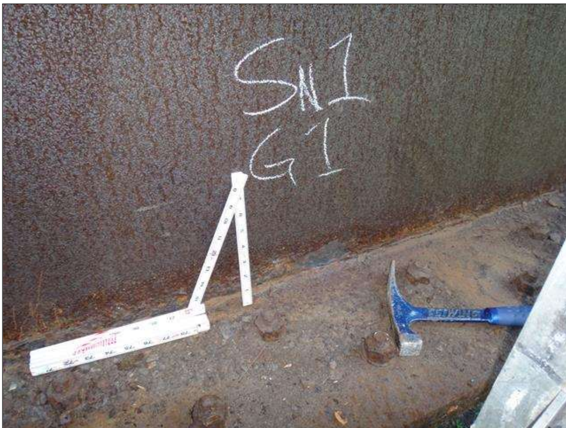
Span 1 Beam 1: along length of exterior face at lower web and web stiffener, active corrosion with section loss [up to 3in high x 1/16in loss]
