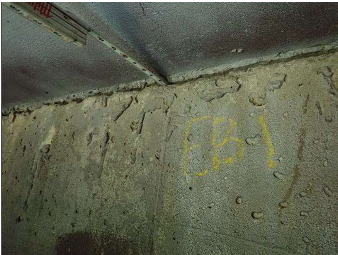
Span 1 Deck: between underside of deck and backwall, gap [up to 3/8in x full length]
