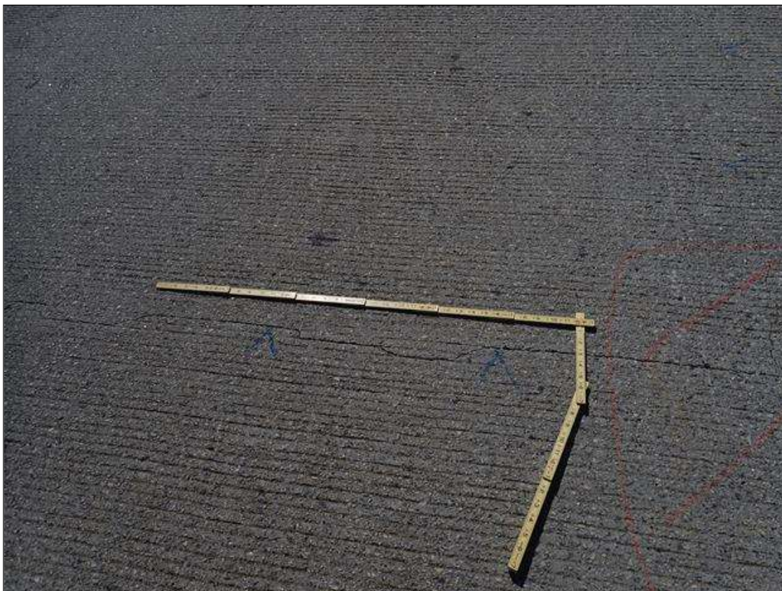
Span 2 Deck: throughout span, multiple transverse cracks [up to full width x 1/16in]
