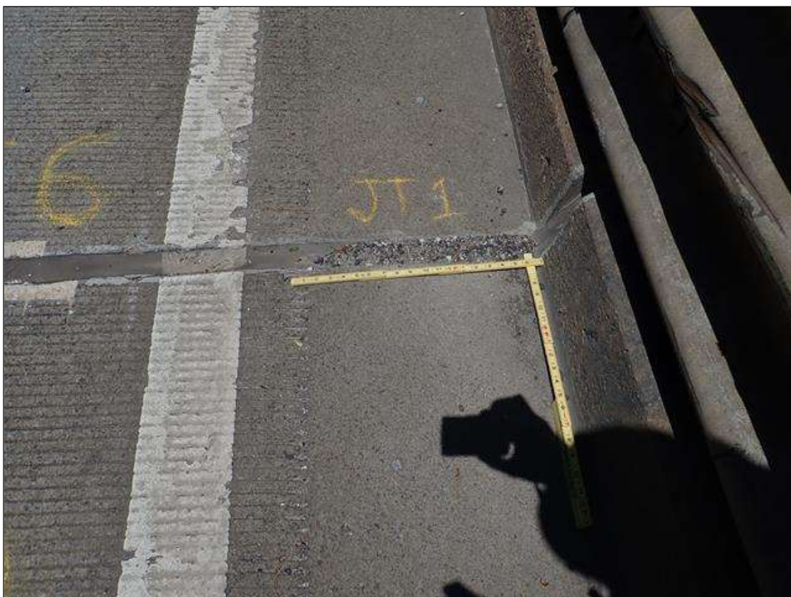
Expansion Joint 1 : at right shoulder, debris accumulation [14in]
