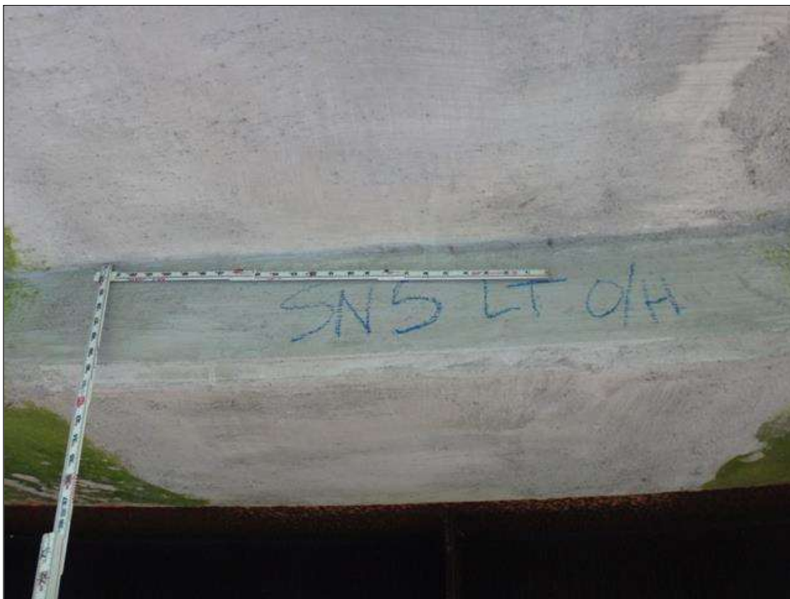
Span 5 Deck: underside West overhang at midspan, sound patch [43in x full width]
