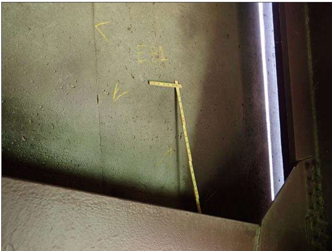
End Bent 1 Abutment/Backwall : left side behind beam 1 bearing, diagonal crack [7ft x up to 0.012in]
