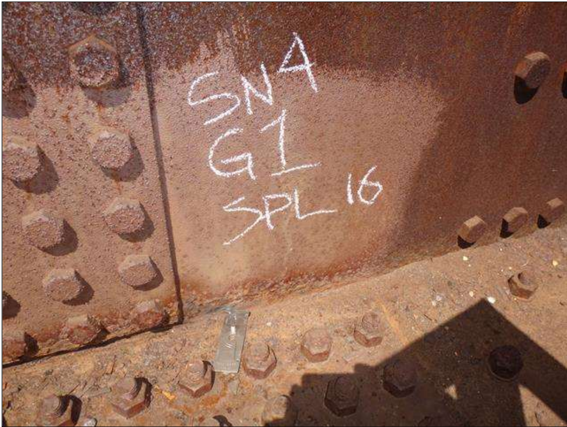
Span 2 Beam 1: [PAR] span 4, interior and exterior face of lower web at splice 16, active corrosion with section loss [4ft x 2in - avg rem 7/16in] with areas of 1/4in loss [avg rem 3/8in]
