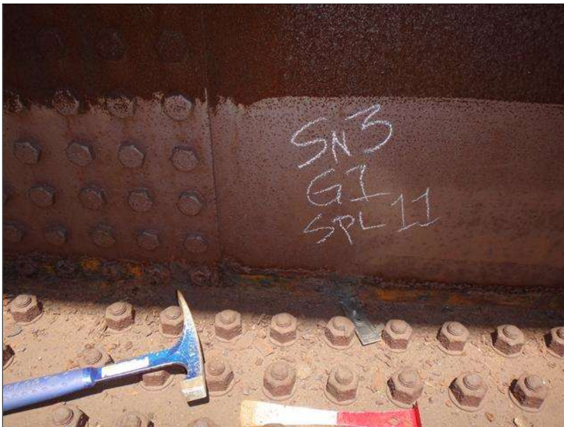
Span 2 Beam 1: span 3, lower web and splice plate both faces at splice plate 11, active corrosion with section loss, web [6.5ft x 3in - avg rem 1/2in] with areas of 3/16in loss [avg rem 3/8in]; plate [full width x 1-1/2in x 1/16in loss], and lower bolts [10% loss]
