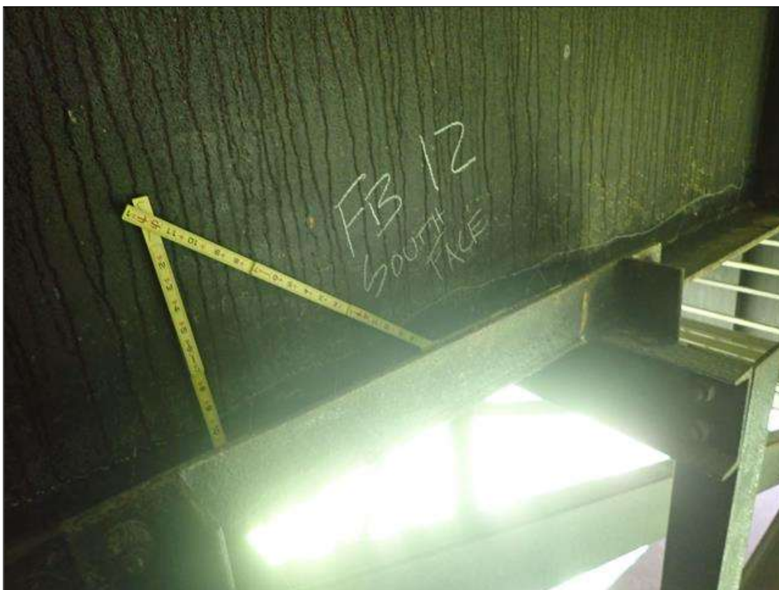
Span 2 Floor Beam 12: [PAR] lower web south face next to girder 1, active corrosion with section loss [7ft x 4in - avg rem 5/16in]
