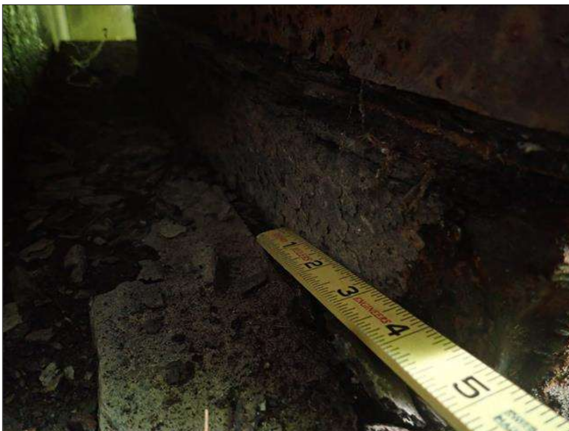
Span 1 Beam 2 Near Bearing: active corrosion with section loss [loss up to 1/8in] with pack rust [1/2in]
