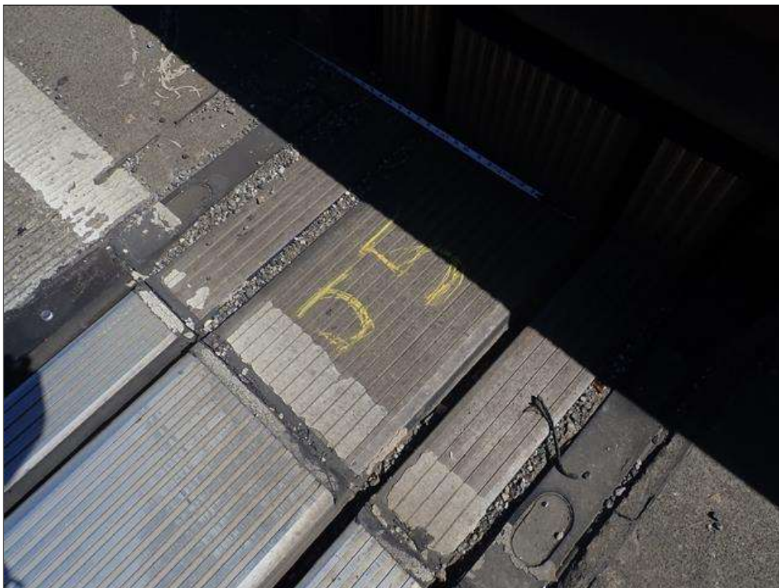
Expansion Joint 2 : at both shoulders, debris accumulation [up to 3ft]
