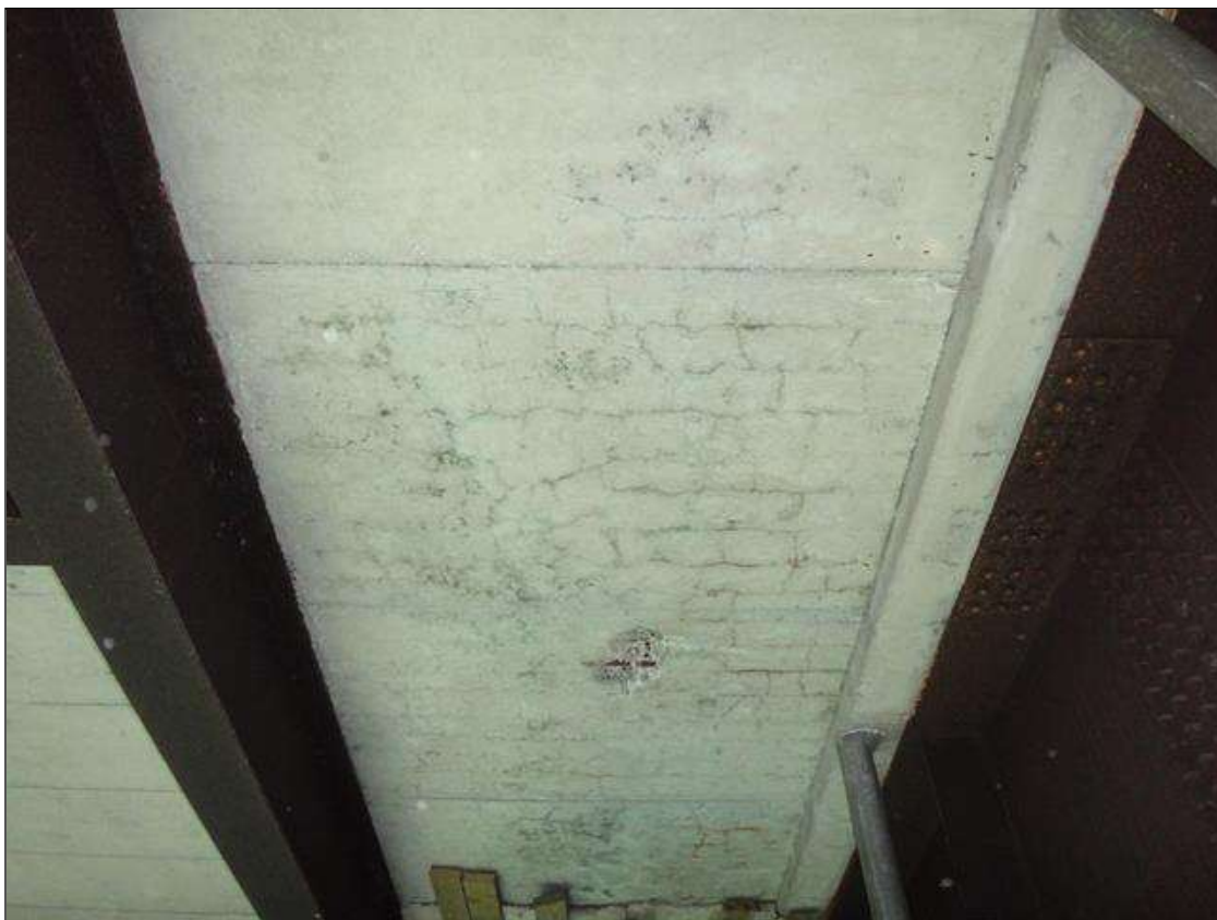
Span 4 Deck: underside of deck at far end, multiple transverse and longitudinal cracks [up to 8ft x 0.03in] with efflorescence and rust stain
