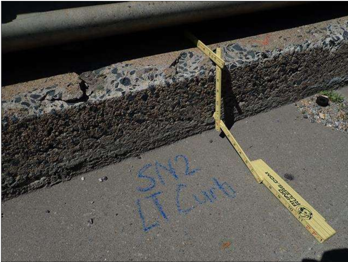
Span 2 Left Bridge Rail: left curb 15ft from joint 5, impact damage [30ft] with spalls [up to 2ft x 5in x 1in deep]
