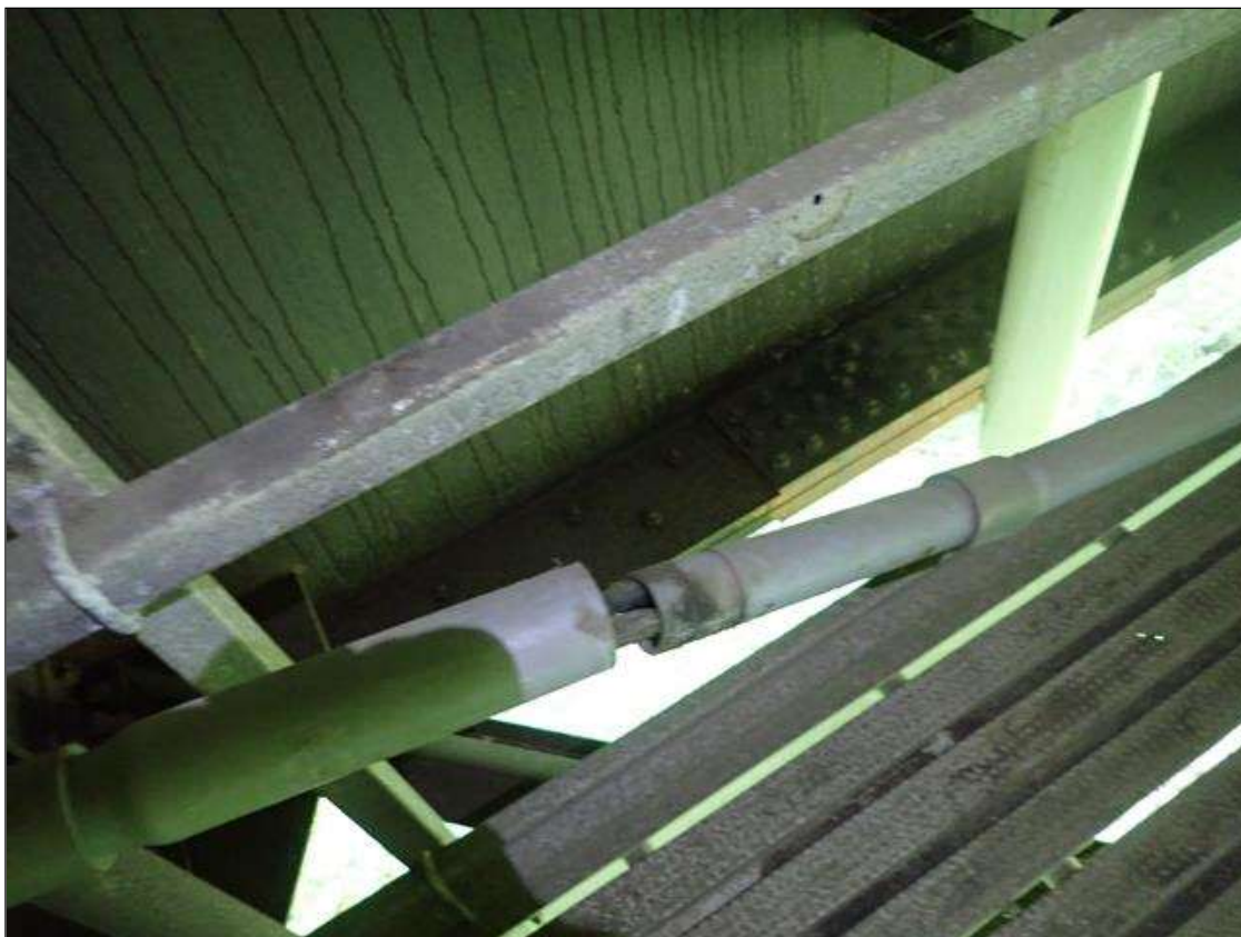
Utilities: span 2 beam 1 between floor beam 3 and 4, attached utility broken and detached
