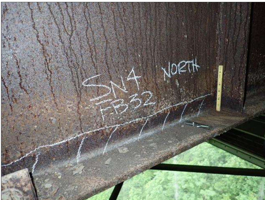
Span 2 Floor Beam 32: lower web North face, active corrosion with section loss [full length x 2in - avg rem 3/8in]
