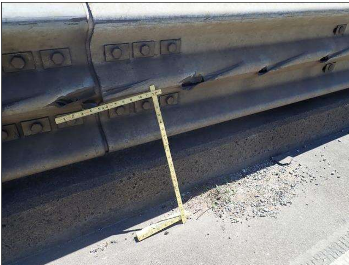
Span 1 Left Bridge Rail: along length of thrie beam, impact damage [full length] with gouges and rips
