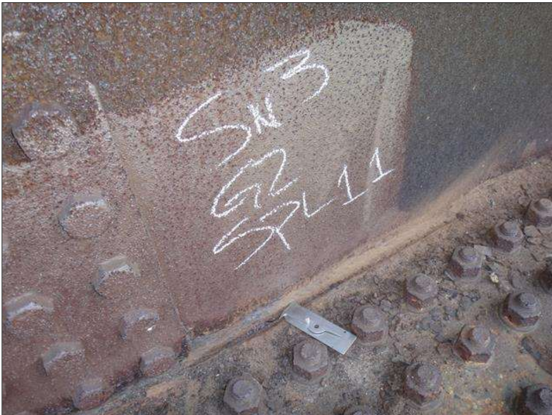
Span 2 Beam 2: span 3, lower web and splice plate exterior face at splice plate 11, active corrosion with section loss, web [7ft-10in x 2in x avg rem 1/2in]; plate [full width x 1-1/2in x 1/16in loss]
