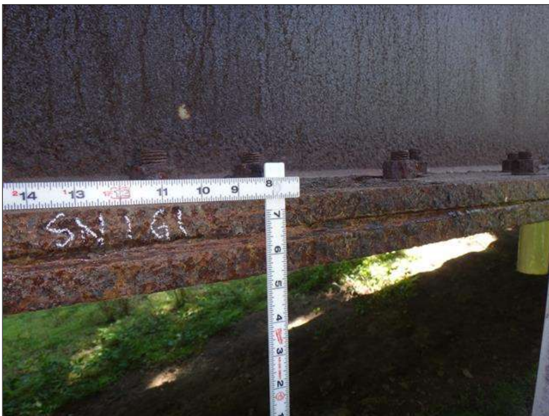
Span 1 Beam 1: along length of bottom flange and cover plate, pack rust [up to 7/16in]
