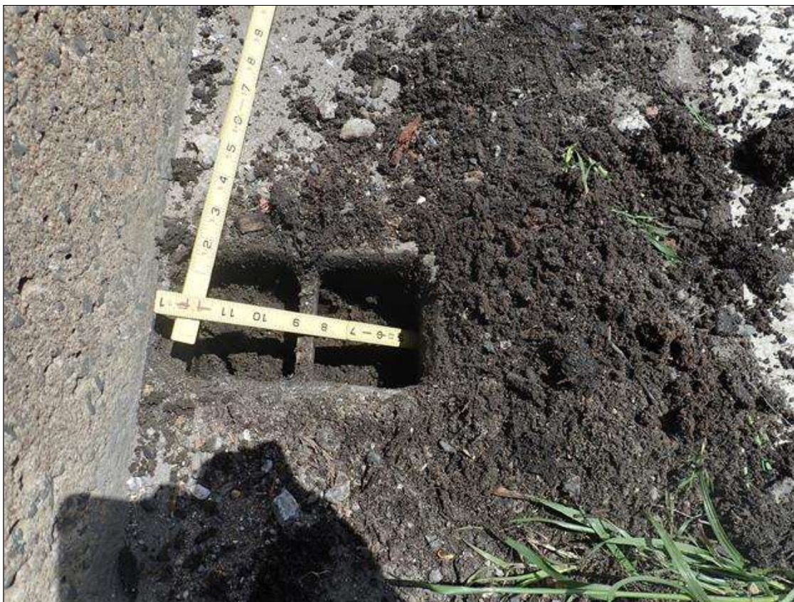
Drainage System: along length of structure, debris accumulation fully blocking drains
