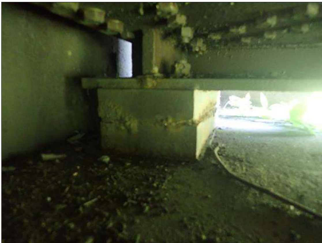
Span 5 Beam 2 Far Bearing: pack rust [up to 1/16in]
