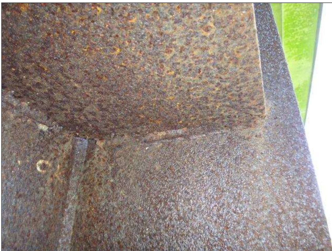
Span 2 Beam 2: poor quality welds found throughout longitudinal and vertical web stiffeners
