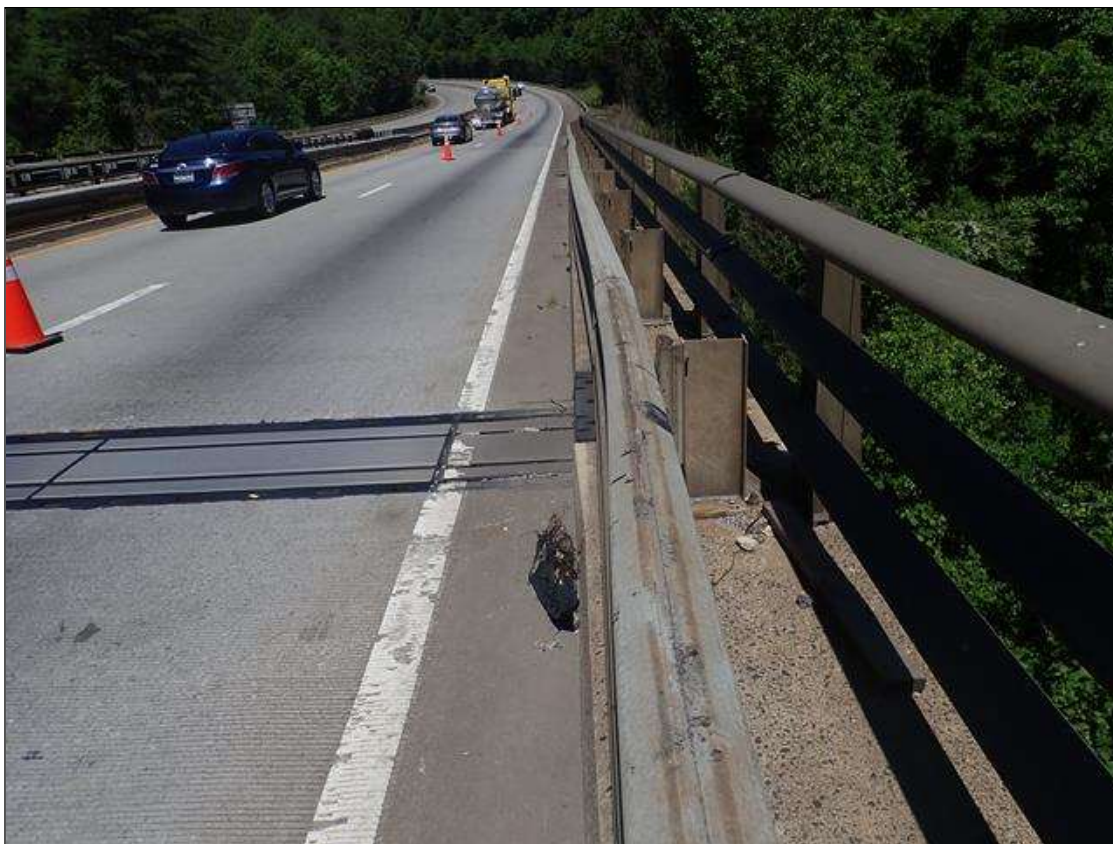
Span 4 Left Bridge Rail: thrie beam at joint 3, impact damage with deflection [45ft x up to 6in deflection]
