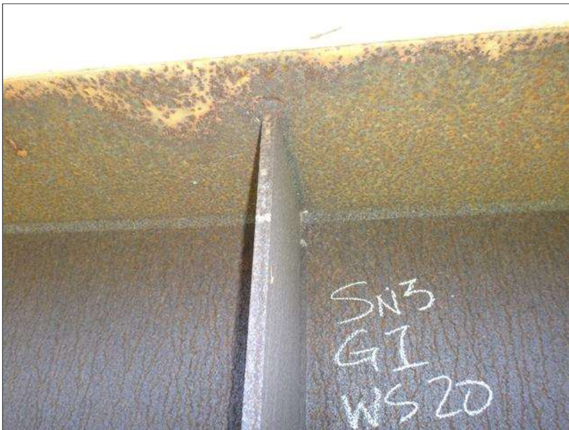
Span 2 Beam 1: exterior face of top flange at web stiffener 20, dye pen test indicates possible 1/8in crack in toe of weld
