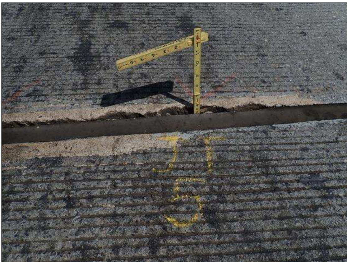
Expansion Joint 6 : along joint, areas of seal adhesion failure [up to 2.5ft x up to full depth]
