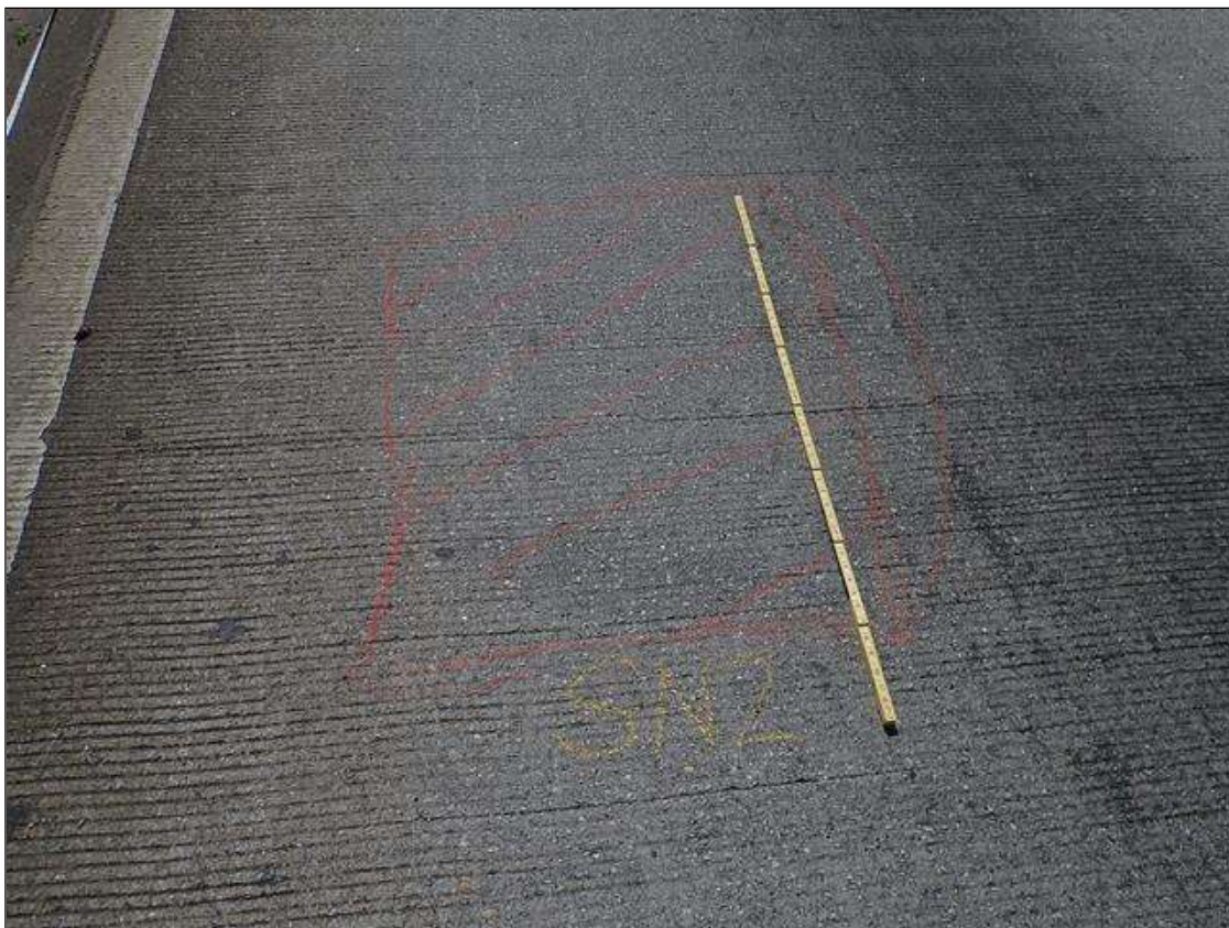
Span 2 Deck: throughout span at random locations, multiple delaminations [up to 7ft x 4ft]
