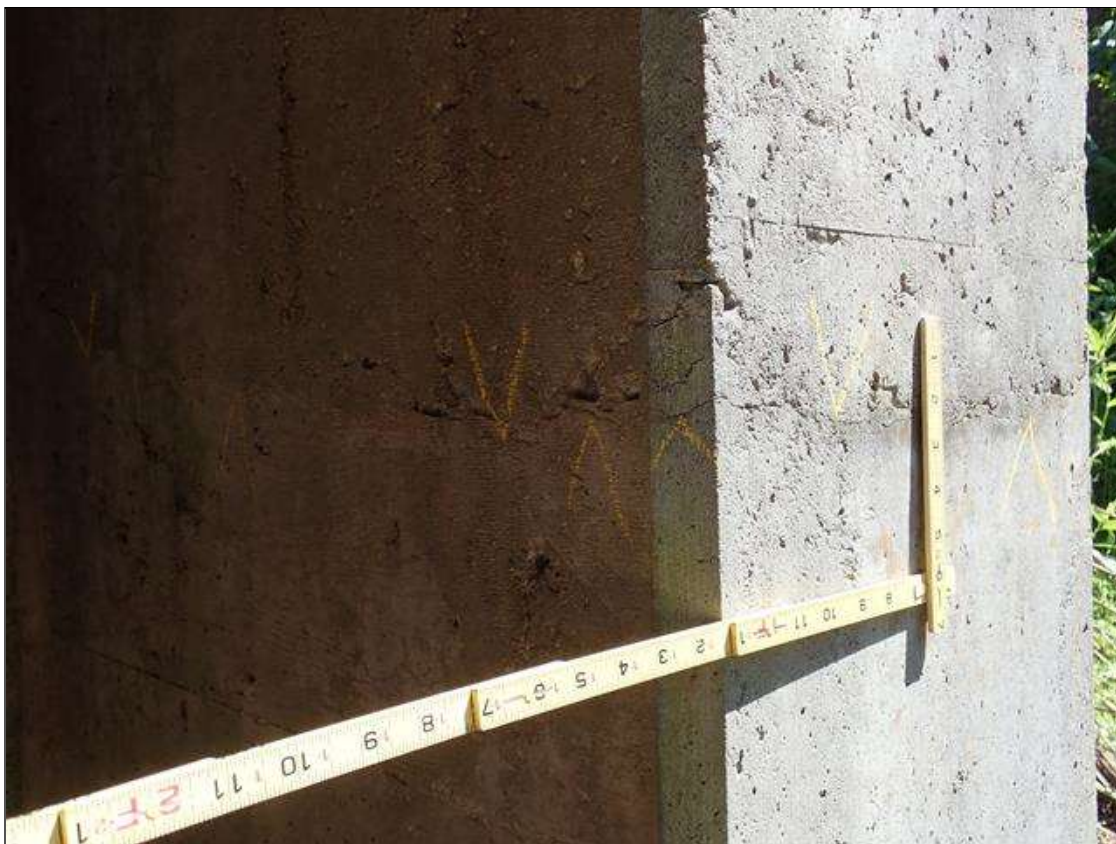
Southwest wingwall: at face of far end and sides, wrap around horizontal crack [4.5ft x up to 0.015in], similar at Southeast wingwall
