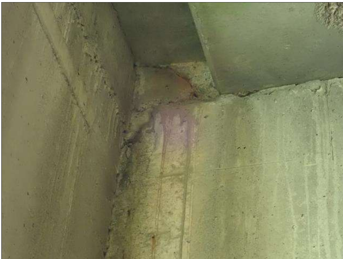
End Bent 1 Abutment/Backwall : top of backwall at right side adjacent to wingwall, spall [9in x 9in x 3in deep], similar at left side
