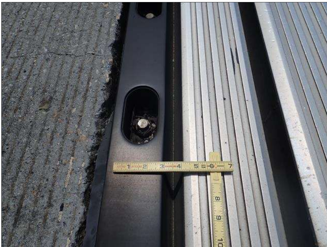
Expansion Joint 5 : both sides of joint, missing plug covers [up to full length]
