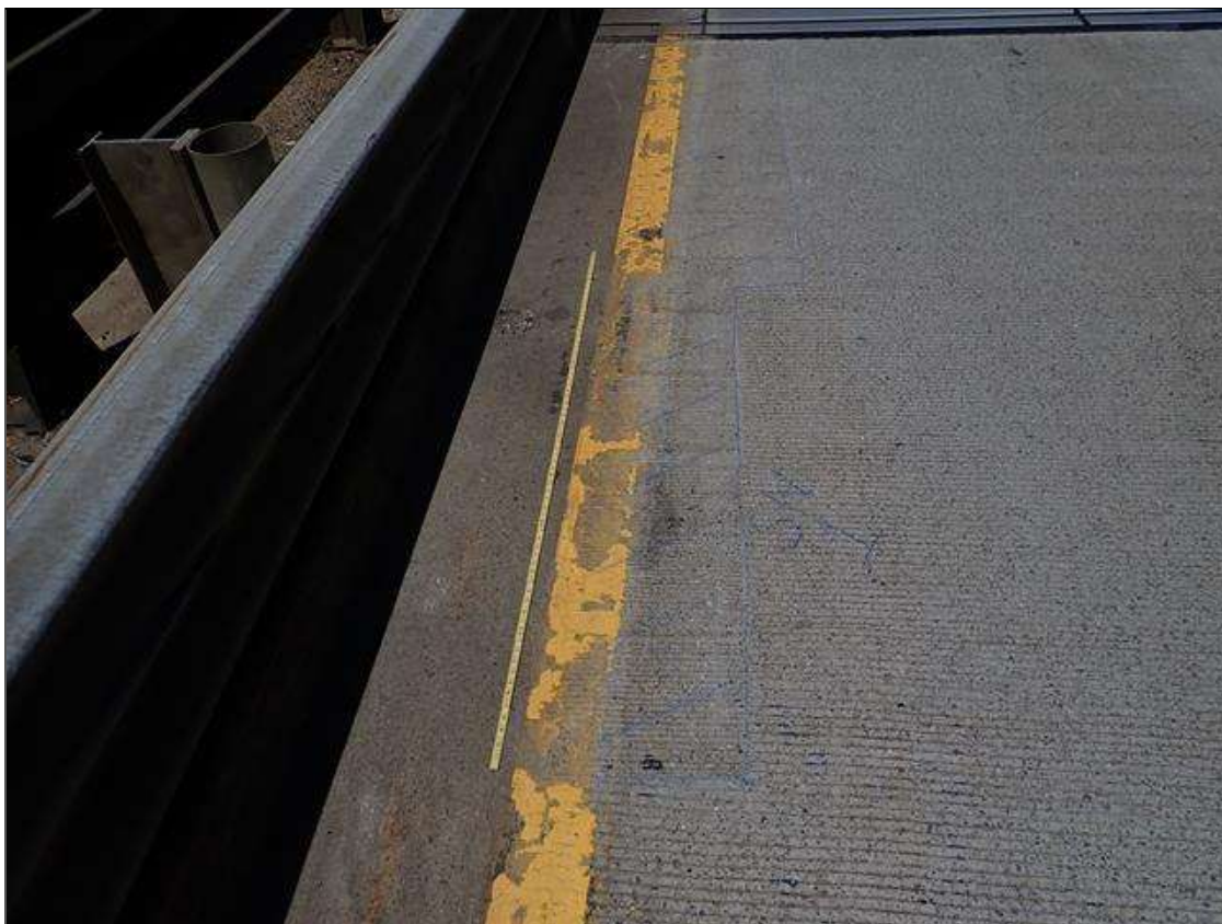
Span 1 Deck: left lane at far end adjacent to yellow line, sound repair [12ft x 1.5ft]
