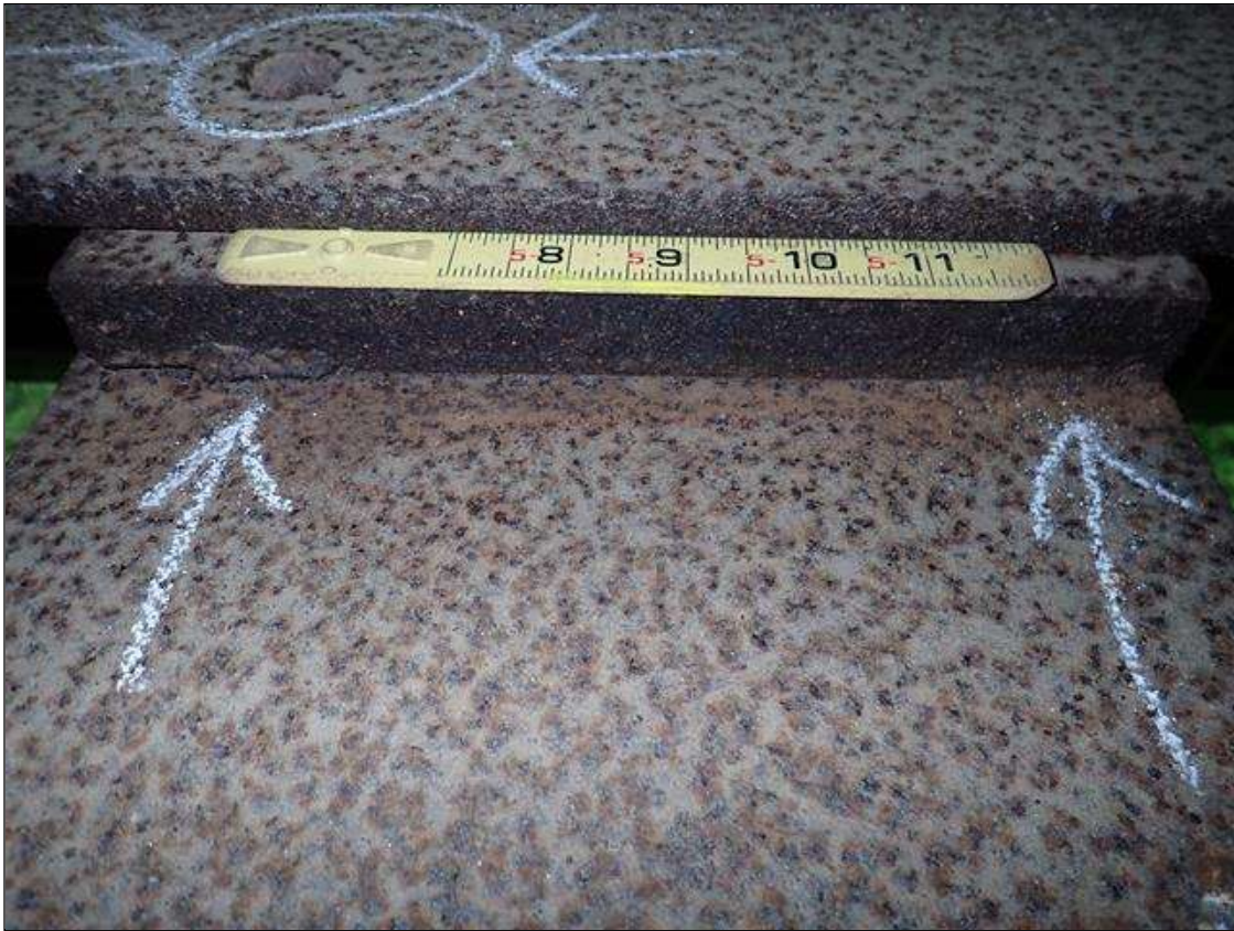
Span 2 Stringer 2: [PAR] at floor beam 33, missing anchor bolts on East face and two cracked tack welds [full length]
