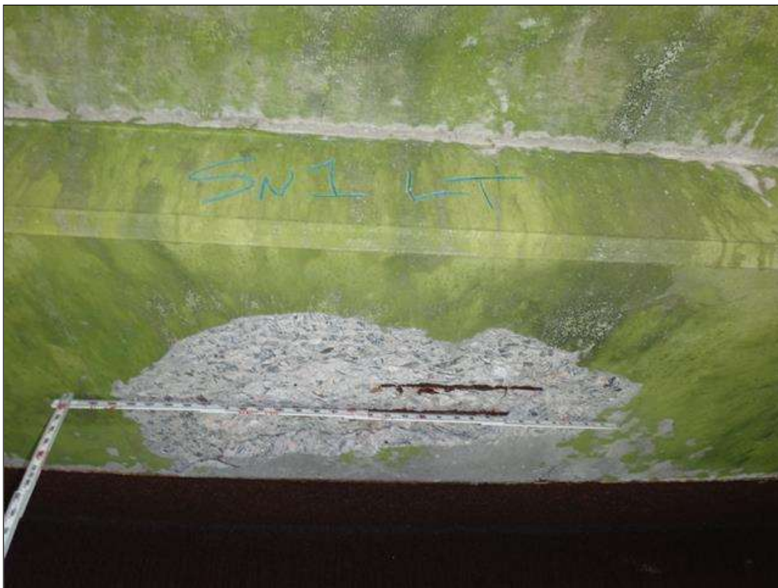
Span 1 Deck: along underside of both overhangs, multiple spalls [up to 29in x 29in x 2in deep] with exposed rusted reinforcing [loss up to 1/16in]
