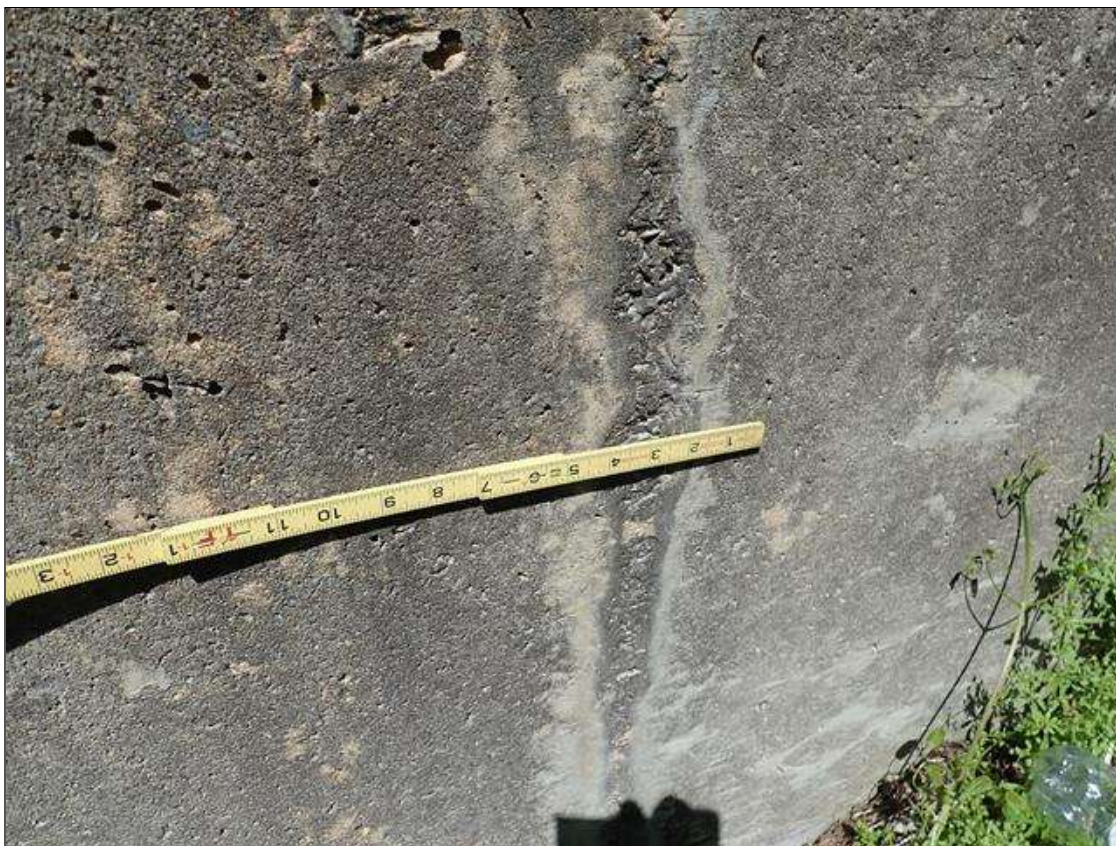
Southwest wingwall: along form lines, exposed coarse aggregate, similar at Southeast wingwall
