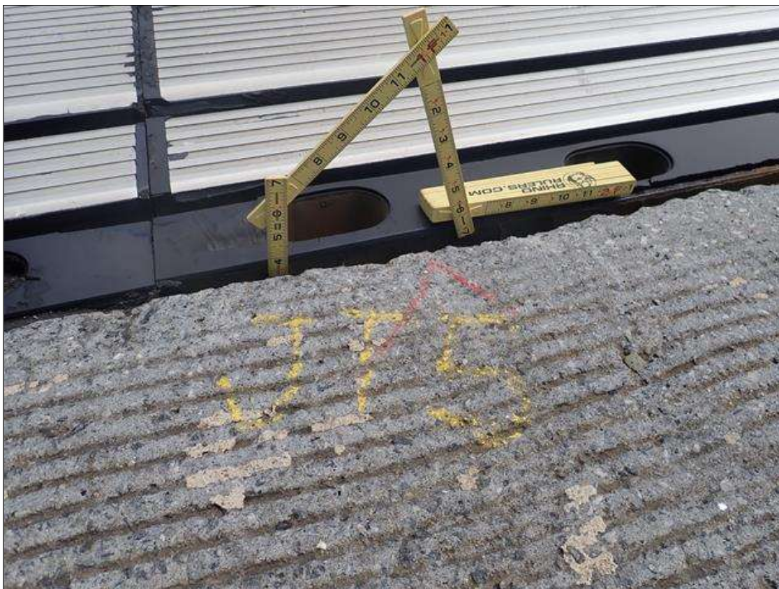
Expansion Joint 5 : along length of joint, missing joint sealant material [up to 20ft] with vertical movement from live load and adjacent edge spalling [up to 12in x 1.5in]
