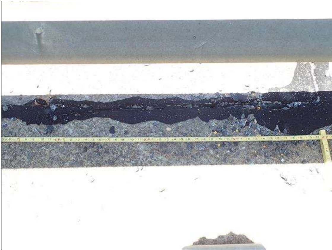
Span 1 Left Bridge Rail: over end bent along joint between wingwall and curb, loss of seal adhesion [up to 4ft] similar at all corners
