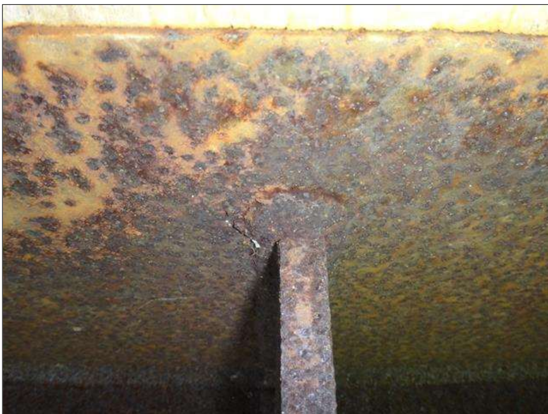
Span 2 Beam 1: exterior face of top flange at web stiffener 20, dye pen test indicates possible 1/8in crack in toe of weld
