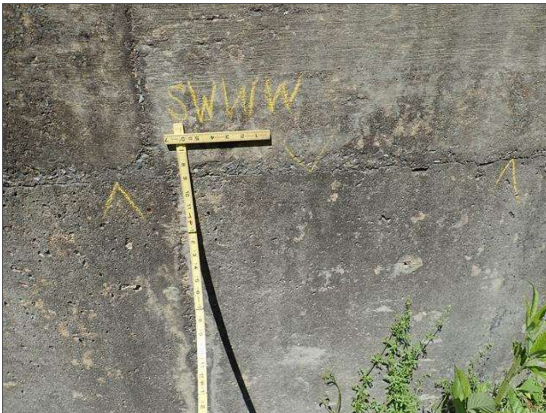
Southwest wingwall: left side 2ft below top edge, horizontal crack [18.5ft x 0.012in]
