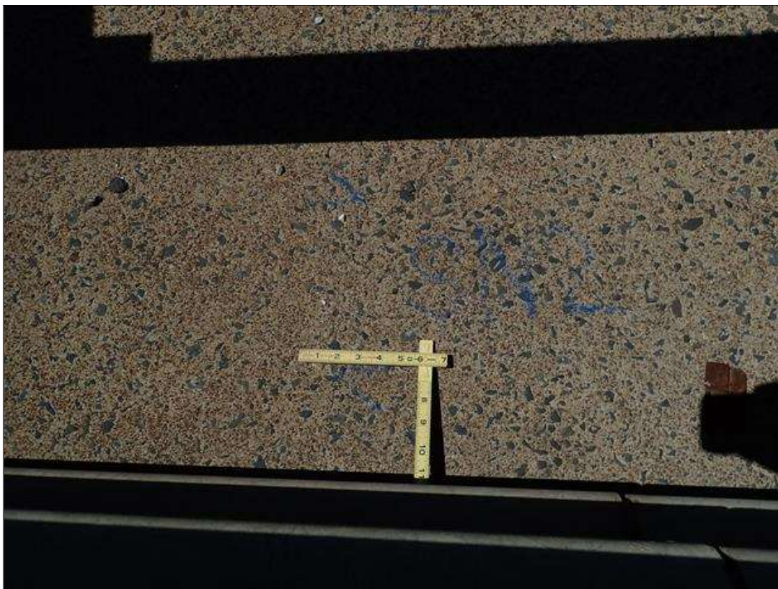
Span 3 Left Bridge Rail: 50ft from bent 3 at curb, transverse crack [full width x 0.012in]
