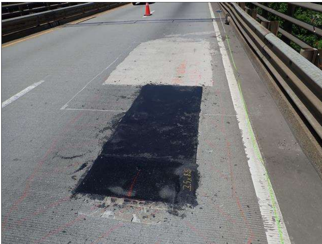
Span 4 Deck: right travel lane at far end, multiple sound patches/repairs [up to 7ft x 12ft]
