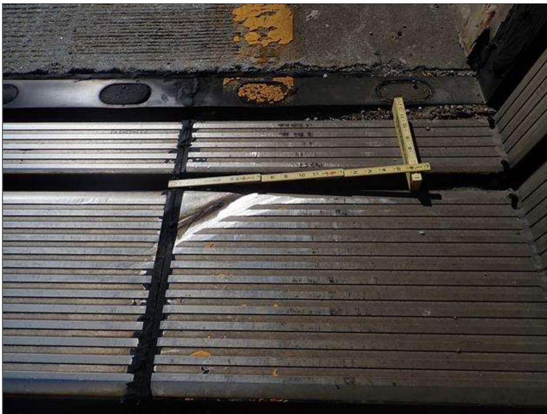
Expansion Joint 2 : in left travel lane at yellow line, damage/gouge [8in x 6in x up to 1/4in deep]
