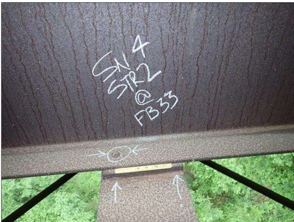
Span 2 Stringer 2: [PAR] at floor beam 33, missing anchor bolts on East face and two cracked tack welds [full length]
