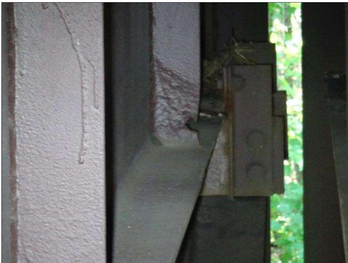
Span 2 Floor Beam 1: first web stiffener from girder 2, painted over pitting [5in x full width x down to knife edge] with corrosion hole [1in diameter]
