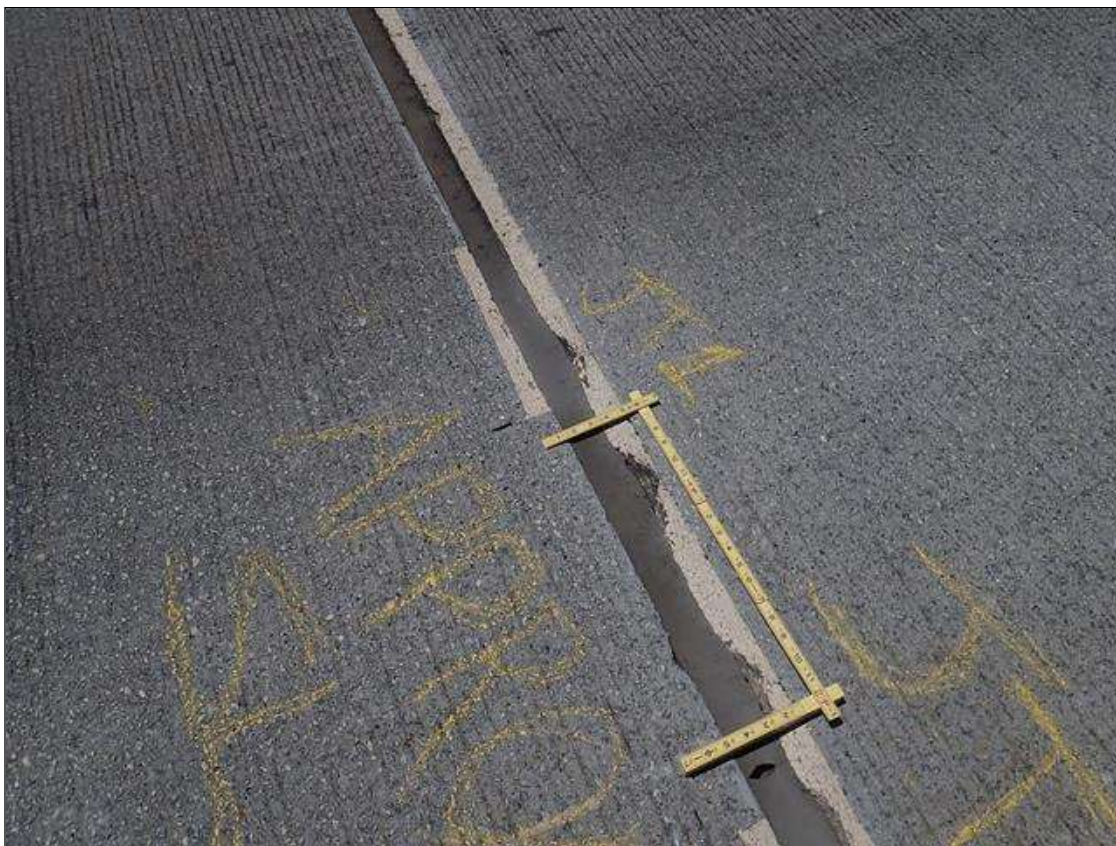
Expansion Joint 1 : at both headers of right lane, multiple edge spalls [up to 6in x 1in x 1in deep] at area of repair
