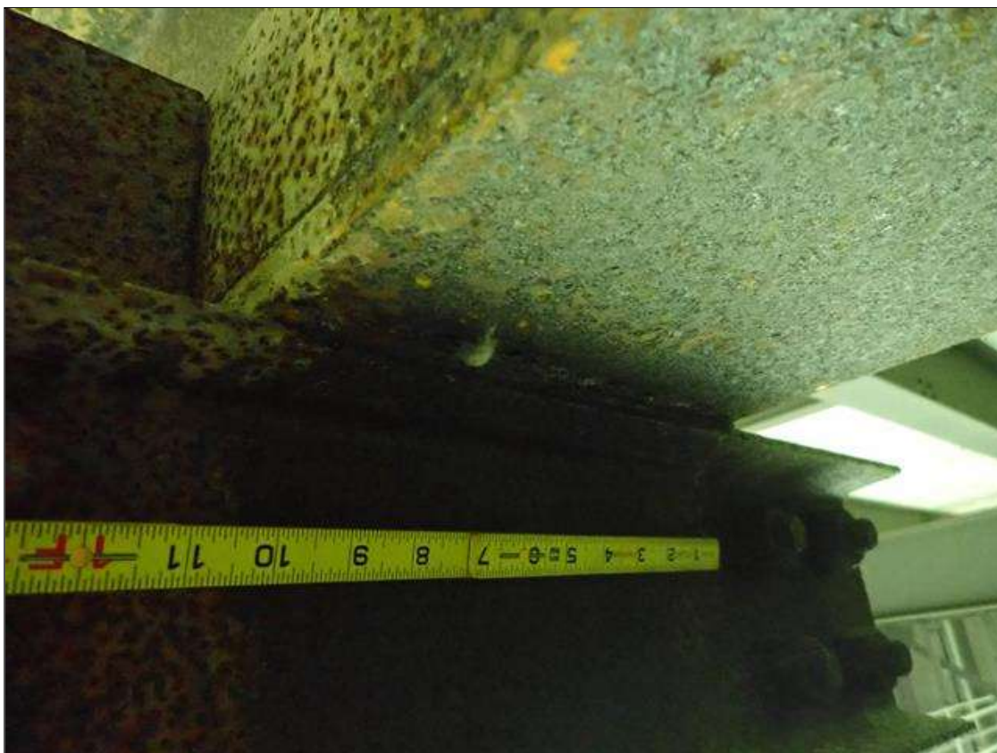
Span 2 Floor Beam 6: underside of bottom flange at catwalk connection, active corrosion with section loss [full width x 1in x up to 1/16in loss]
