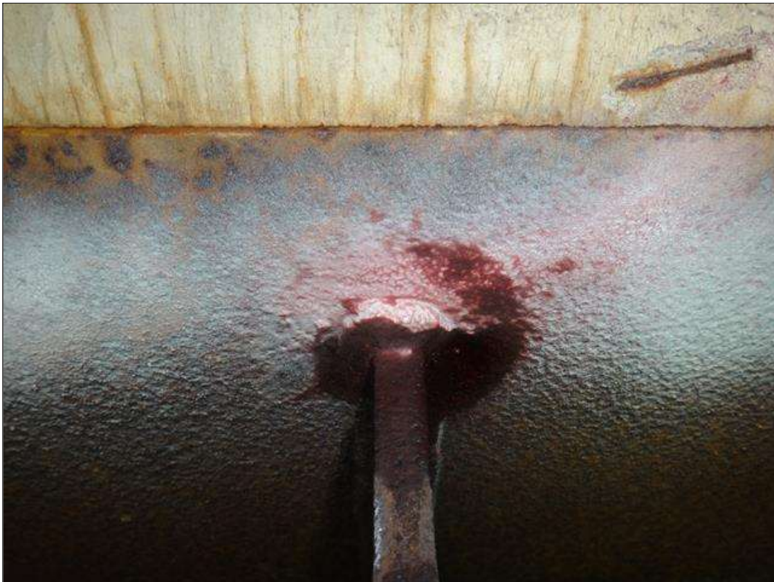
Span 2 Beam 1: exterior face of top flange at web stiffener 20, dye pen test indicates possible 1/8in crack in toe of weld
