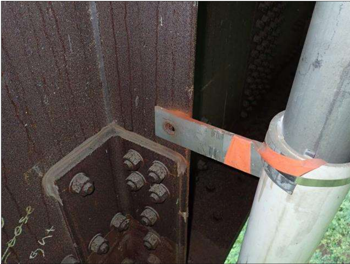
Drainage System: girder 2 downspout South of floor beam 8, lower connection bolt missing
