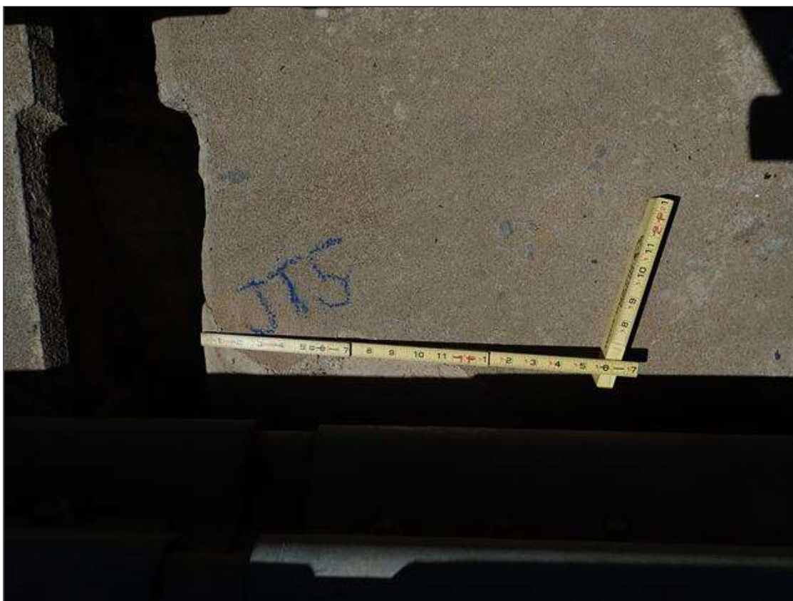
Span 5 Left Bridge Rail: curb adjacent to joint 5, sound patches [up to 14in x up to 12in x up to 9in]
