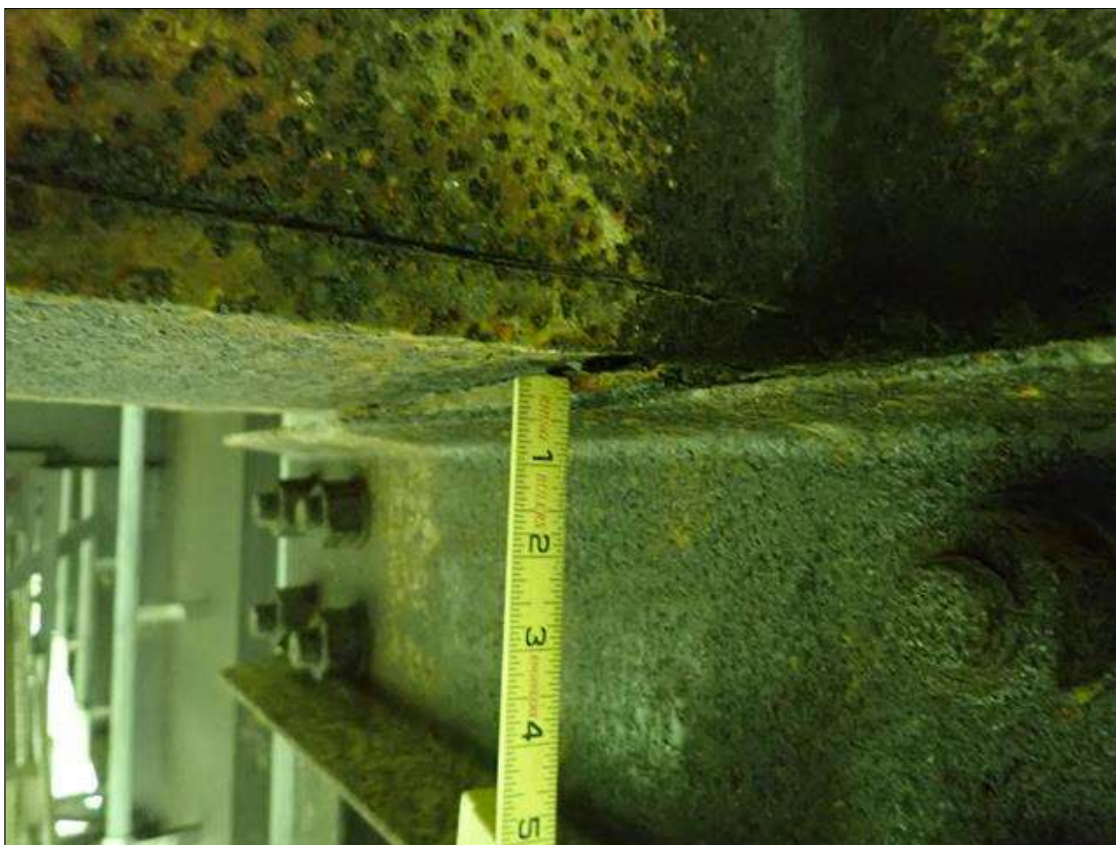
Span 2 Floor Beam 6: between floor beam bottom flange and catwalk hanger at girder 1, pack rust [1/8in] with section loss [up to 1/16in]
