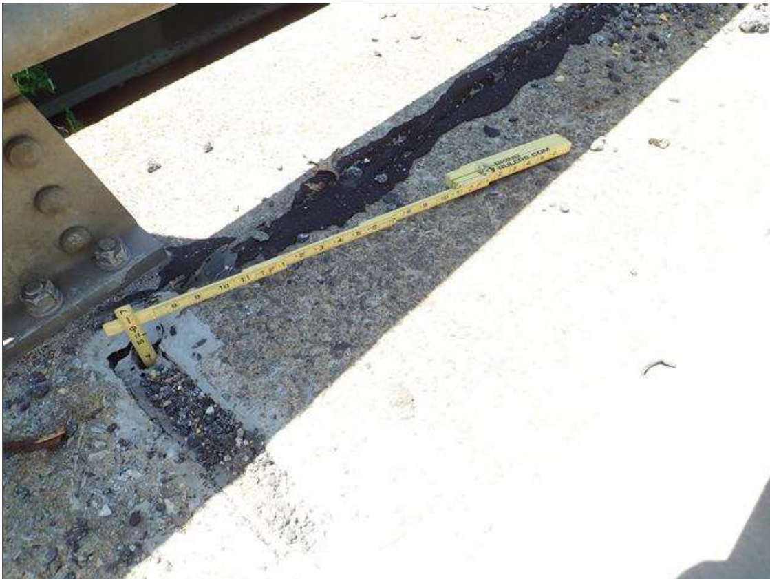
Span 1 Left Bridge Rail: over end bent along joint between wingwall and curb, loss of seal adhesion [up to 4ft] similar at all corners
