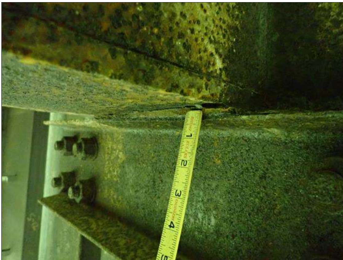
Span 2 Floor Beam 6: between floor beam bottom flange and catwalk hanger at girder 1, pack rust [1/8in] with section loss [up to 1/16in]
