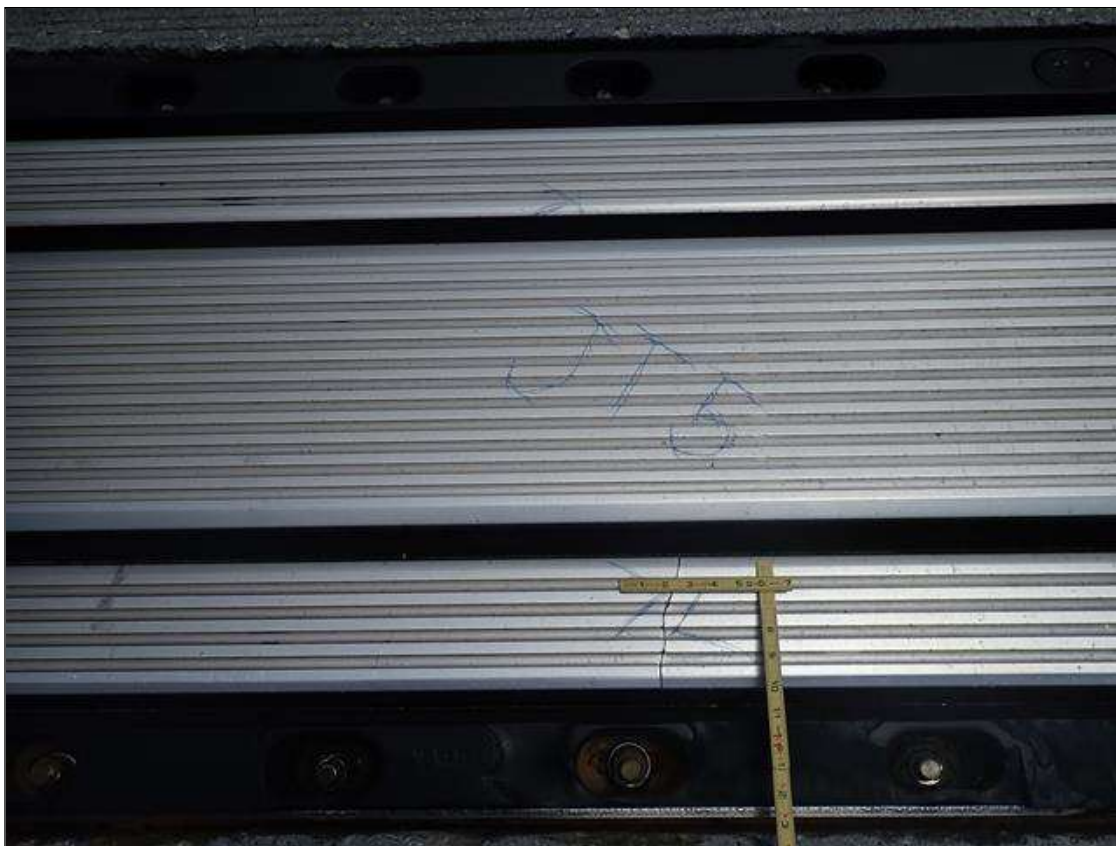
Expansion Joint 5 : [PAR] right travel lane left wheel path in aluminum, two [2] cracks [up to 5in x up to 1/16in]
