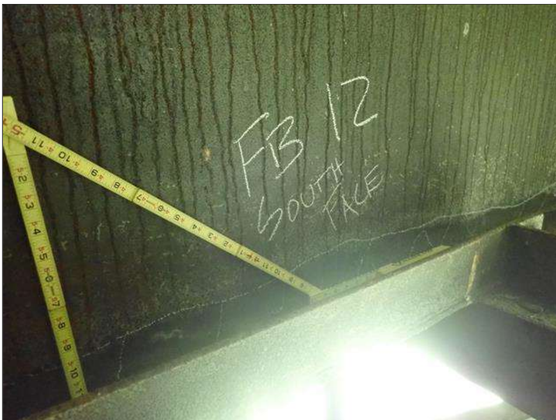
Span 2 Floor Beam 12: [PAR] lower web south face next to girder 1, active corrosion with section loss [7ft x 4in - avg rem 5/16in]
