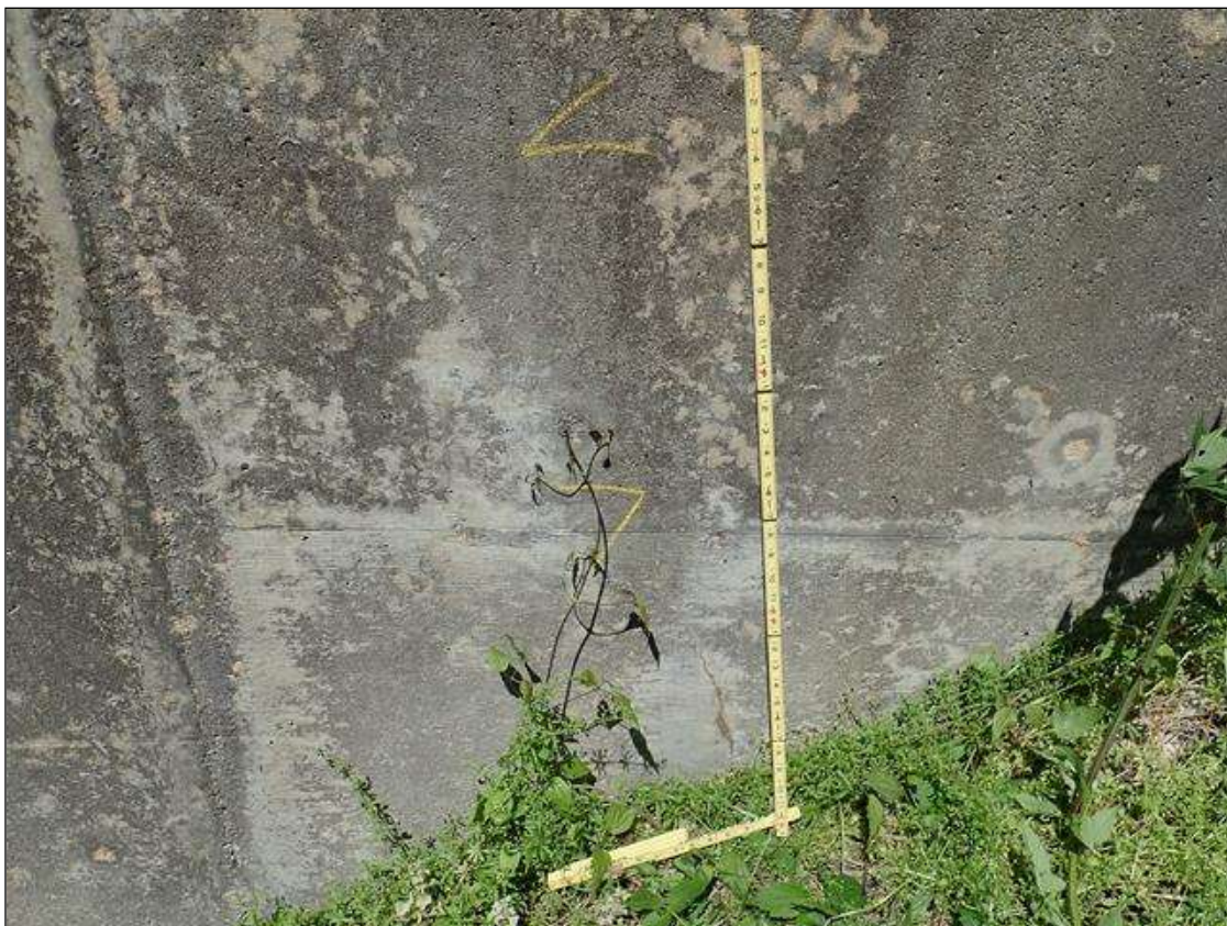
Southwest wingwall: left side 9ft from far end, vertical crack [5ft x hairline] with efflorescence
