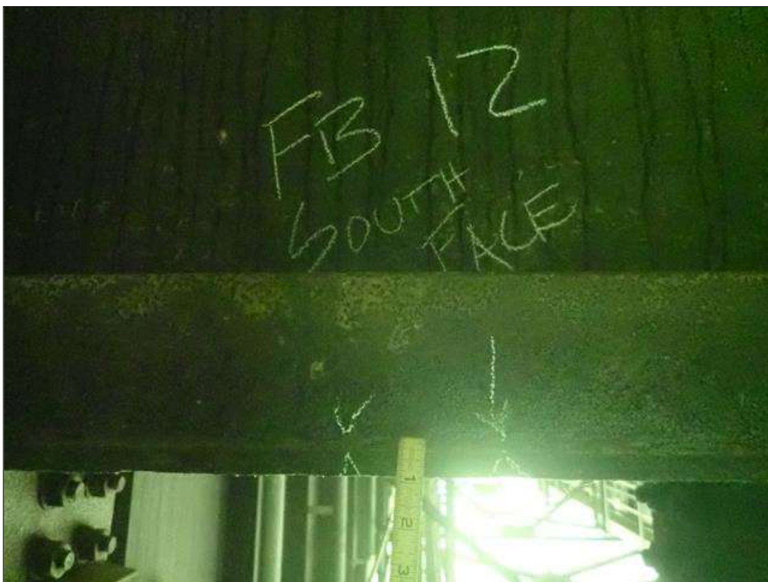
Span 2 Floor Beam 12: between floor beam bottom flange and catwalk hanger at both girders, pack rust [up to 1/4in]
