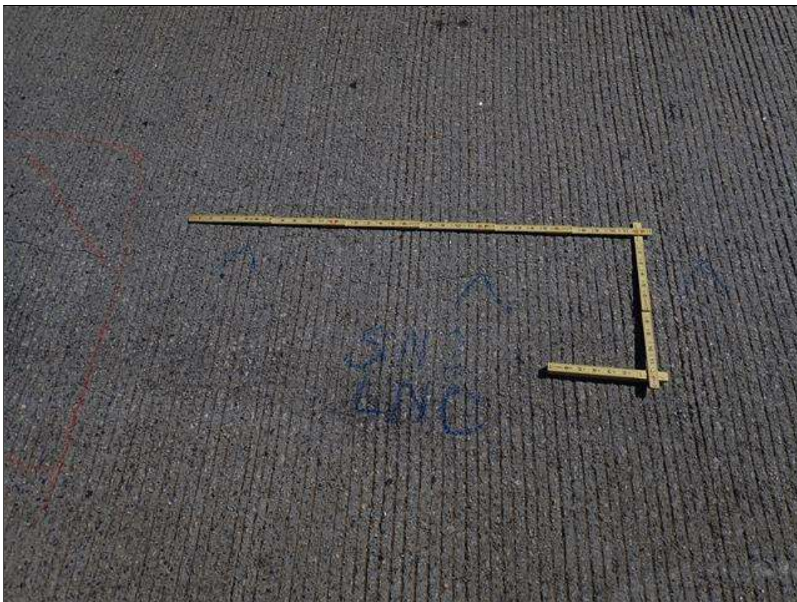
Span 2 Deck: throughout span, multiple longitudinal cracks [up to 30ft x 0.03in]
