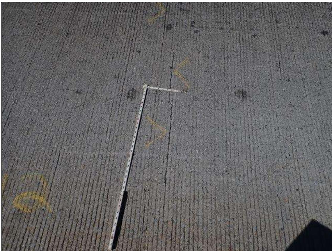
Span 2 Deck: throughout span, multiple transverse cracks [up to full width x 1/16in]
