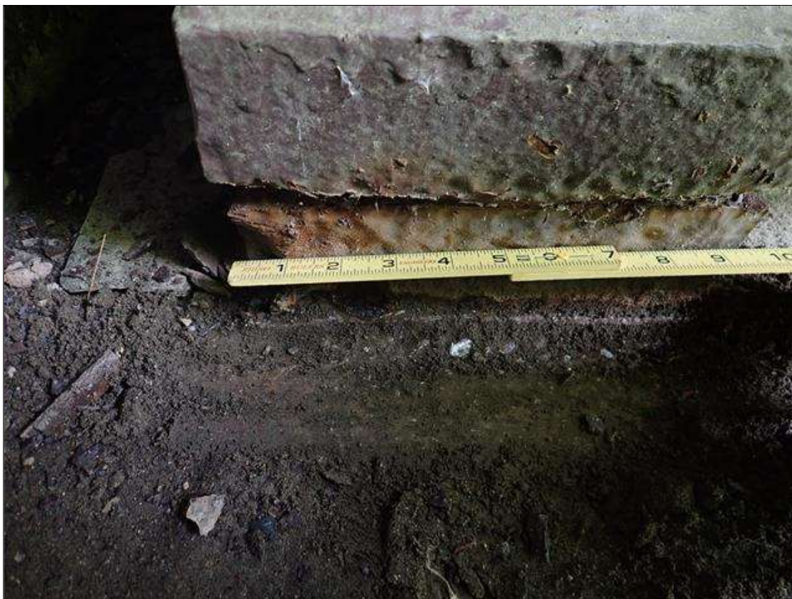
Span 1 Beam 2 Near Bearing: active corrosion with section loss [loss up to 1/8in] with pack rust [1/2in]
