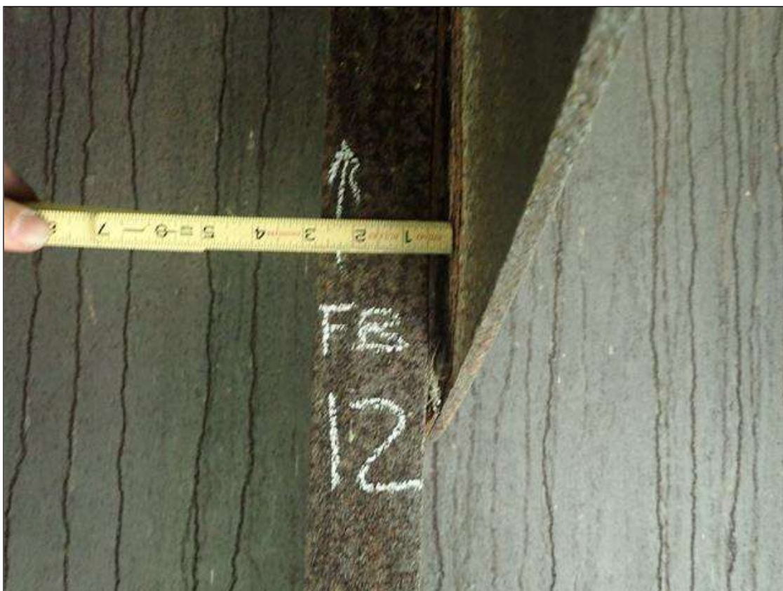
Span 2 Floor Beam 12: between upper gusset plate and web stiffener at both girders, pack rust [up to 1/2in]
