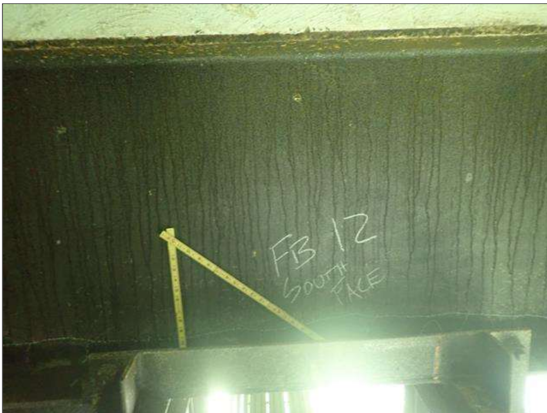
Span 2 Floor Beam 12: [PAR] lower web south face next to girder 1, active corrosion with section loss [7ft x 4in - avg rem 5/16in]
