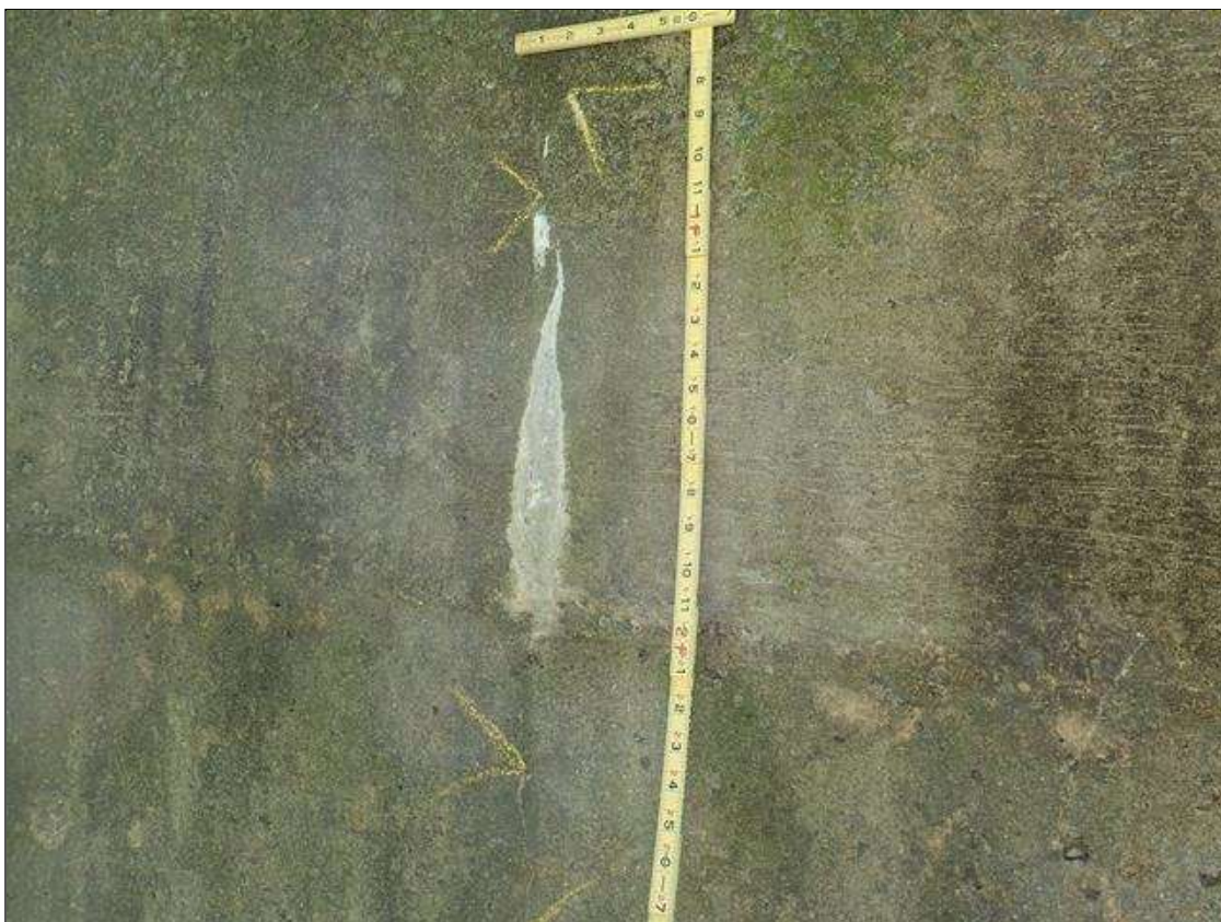
Southeast wingwall: right face at far end and mid length, two [2] vertical cracks [up to 3t x hairline] with efflorescence build-up
