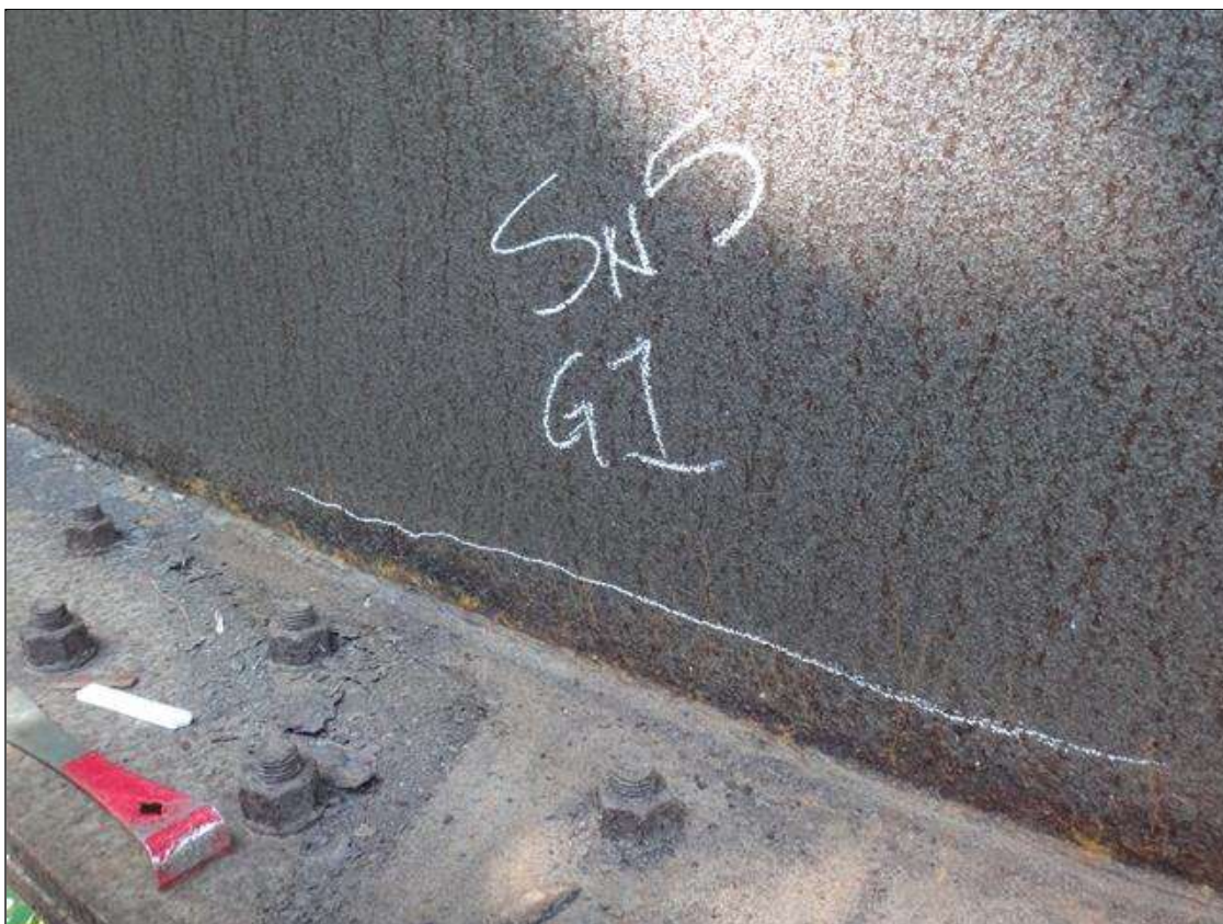
Span 1 Beam 2: lower web along length of exterior face, active corrosion with section loss [85ft x up to 2-1/2in x up to 3/32in deep]
