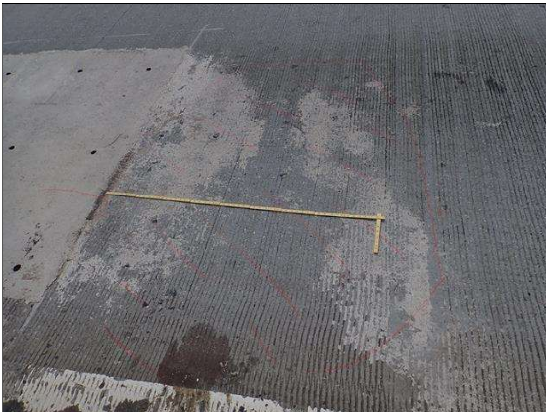
Span 4 Deck: adjacent to repairs at far end, multiple delaminations [up to 5.5ft x 7ft]
