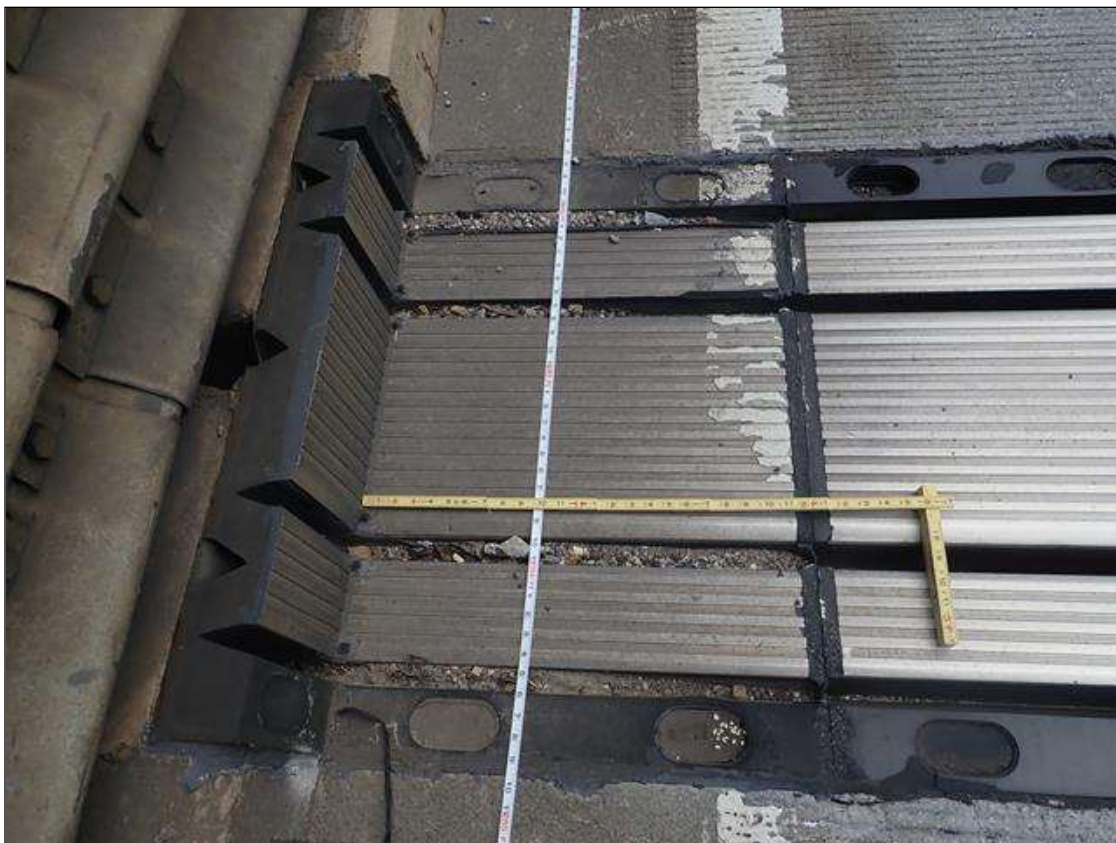
Expansion Joint 5 : at both shoulders, debris accumulation [up to 18in]
