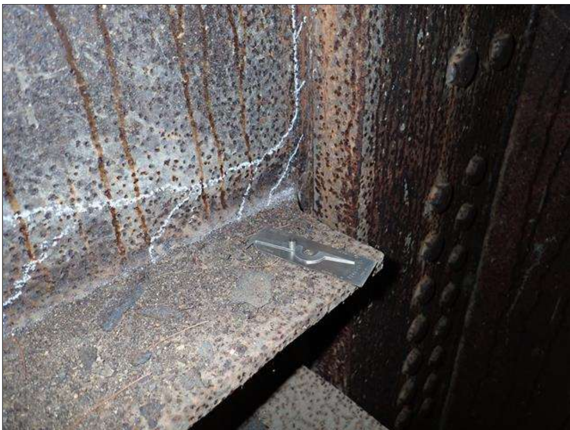
Span 2 Floor Beam 12: lower web South face next to girder 2, active corrosion with section loss [full height x up to 2in - avg rem 3/8in] with pack rust [up to 5/16in]
