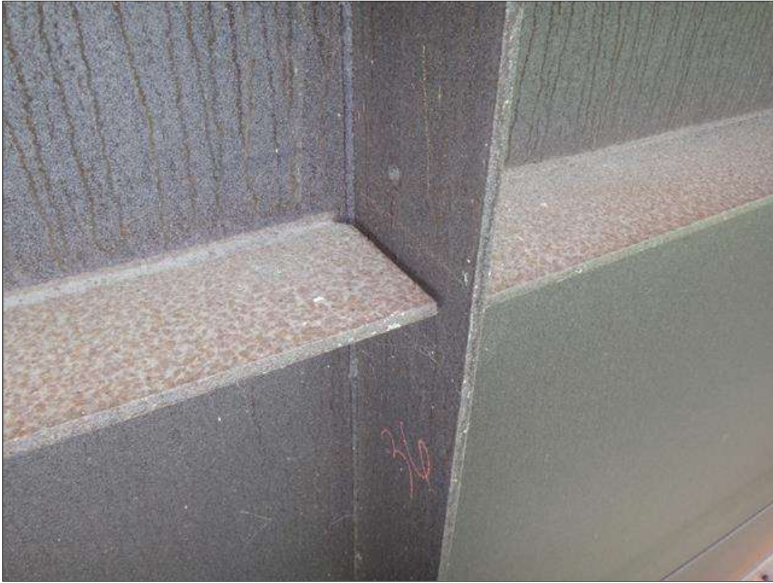
Span 2 Beam 2: span 4, exterior face at web stiffener 36, no weld between horizontal and vertical stiffener [both sides], similar at stiffener 37
