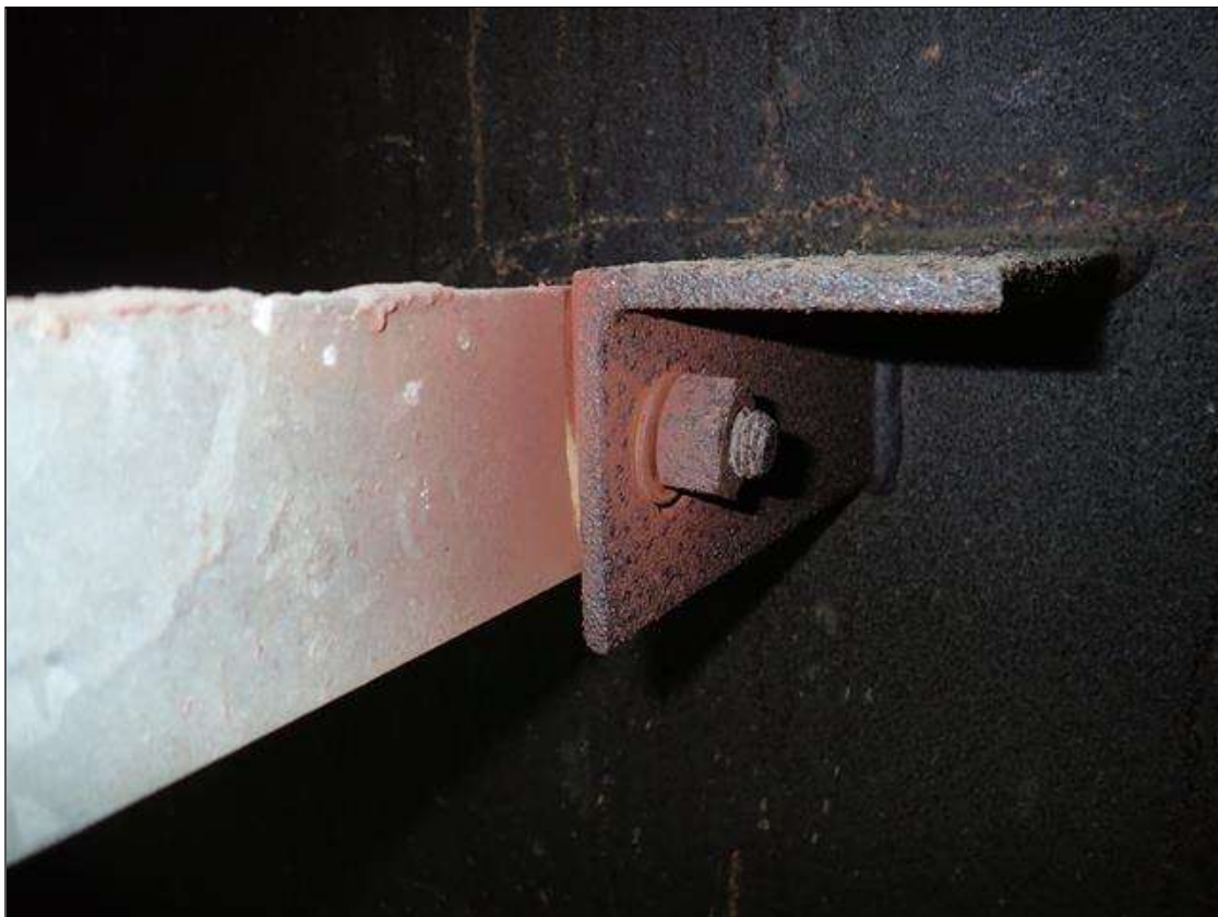
Drainage System: girder 2 downspout South of floor beam 7, loose bottom connection bolt with fretting rust
