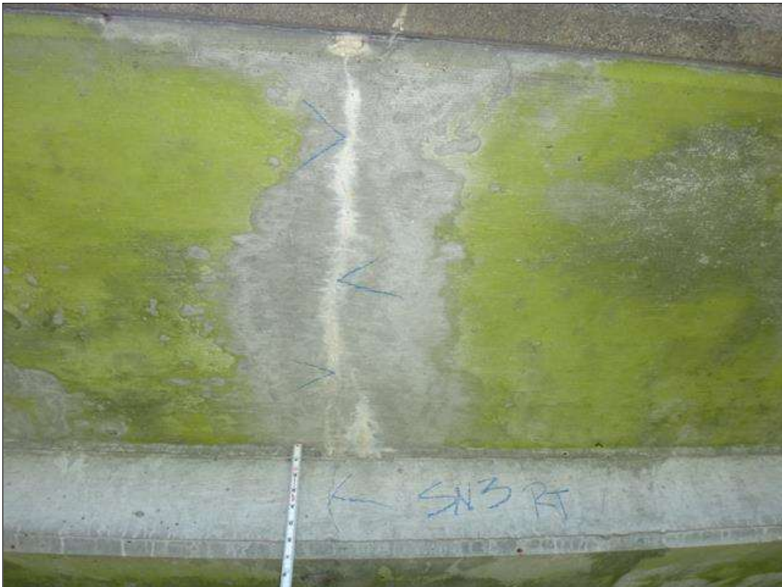
Span 2 Deck: underside East overhang scattered throughout, multiple transverse cracks [full width x hairline] with efflorescence, West overhang similar
