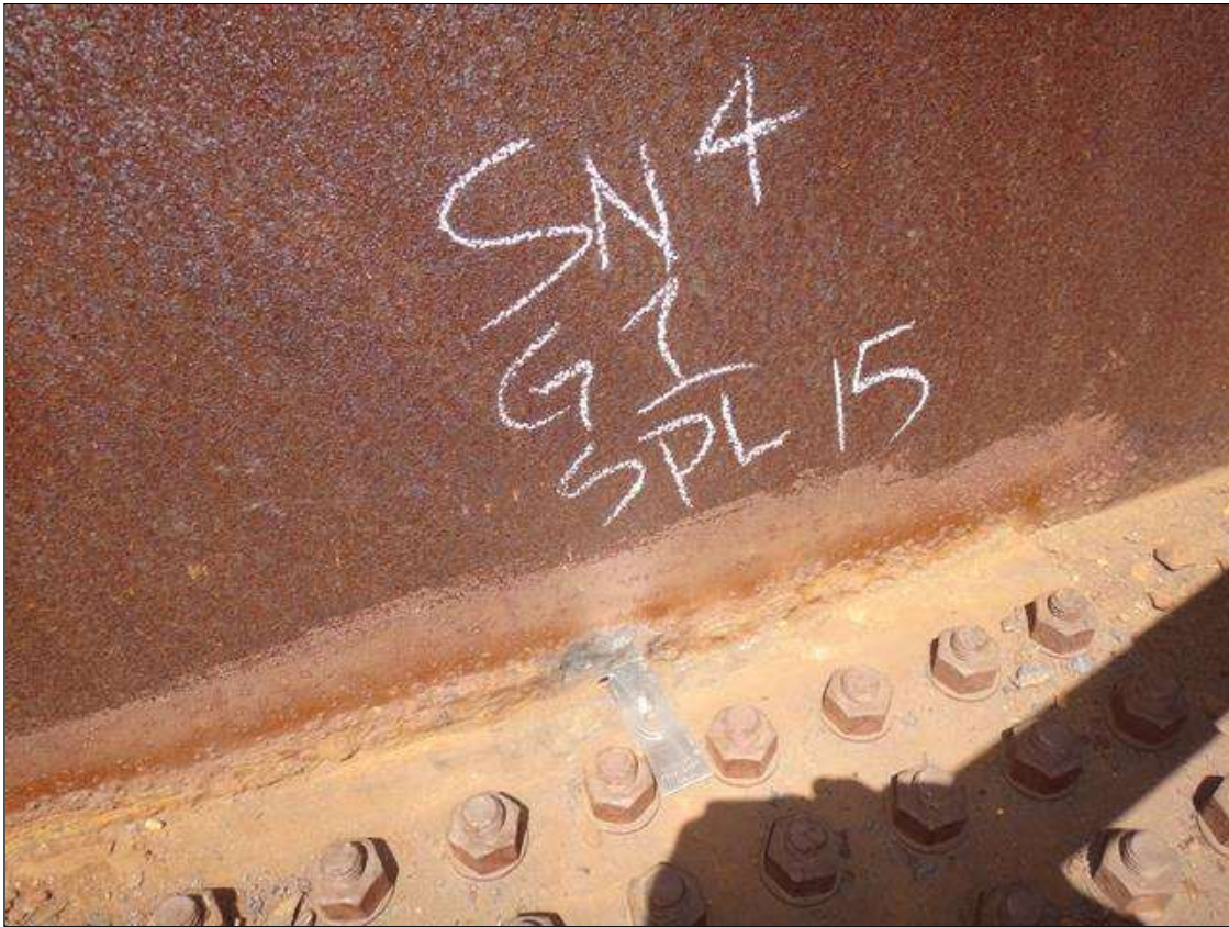
Span 2 Beam 1: span 4, lower web and splice plate exterior face at splice plate 16, active corrosion with section loss, web [4ft x 2in - avg rem 7/16in]; top of plate [full width x 1in x 1/16in loss]
