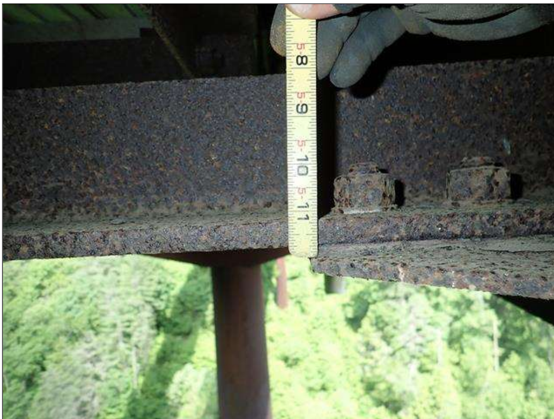
Span 2 Beam 2: span 2, between connection plate and lateral bracing at floor beam 9, pack rust [up to 3/16in]
