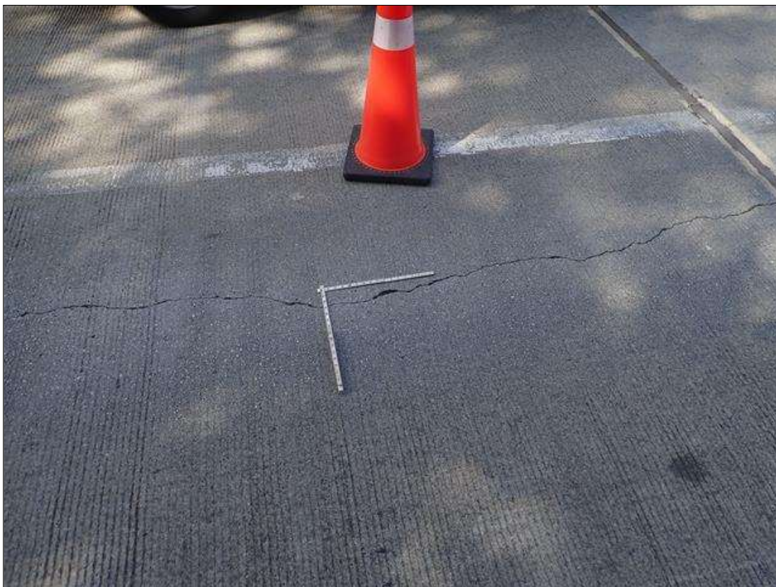
Approach 1: Northbound right lane at center, longitudinal crack [full length x 1/8in]
