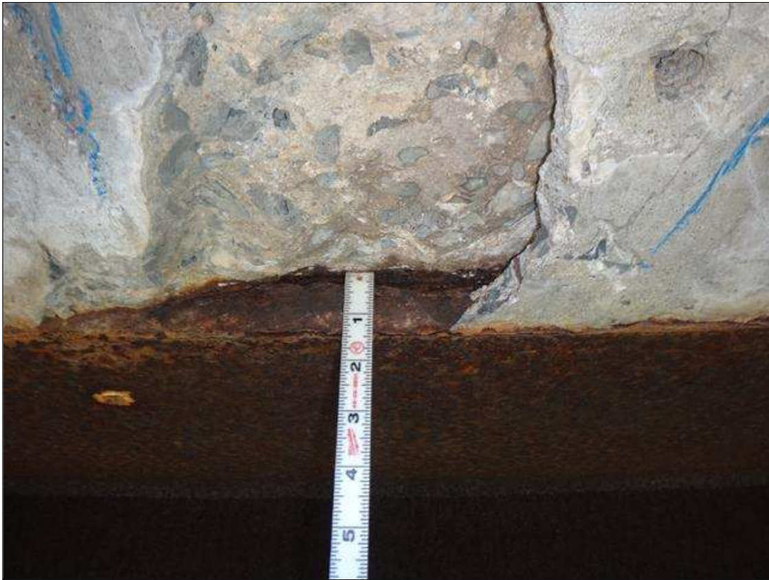
Span 3 Deck: underside left overhang at web stiffener 21, spall/delamination [7ft-10in x 13in x 1-1/4in deep] with pack rust between top flange and deck [1/4in]
