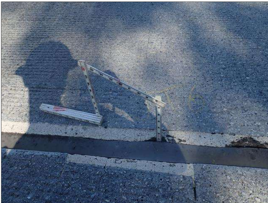
Expansion Joint 1 : along joint in right lane, seal adhesion failure [up to 2in deep]
