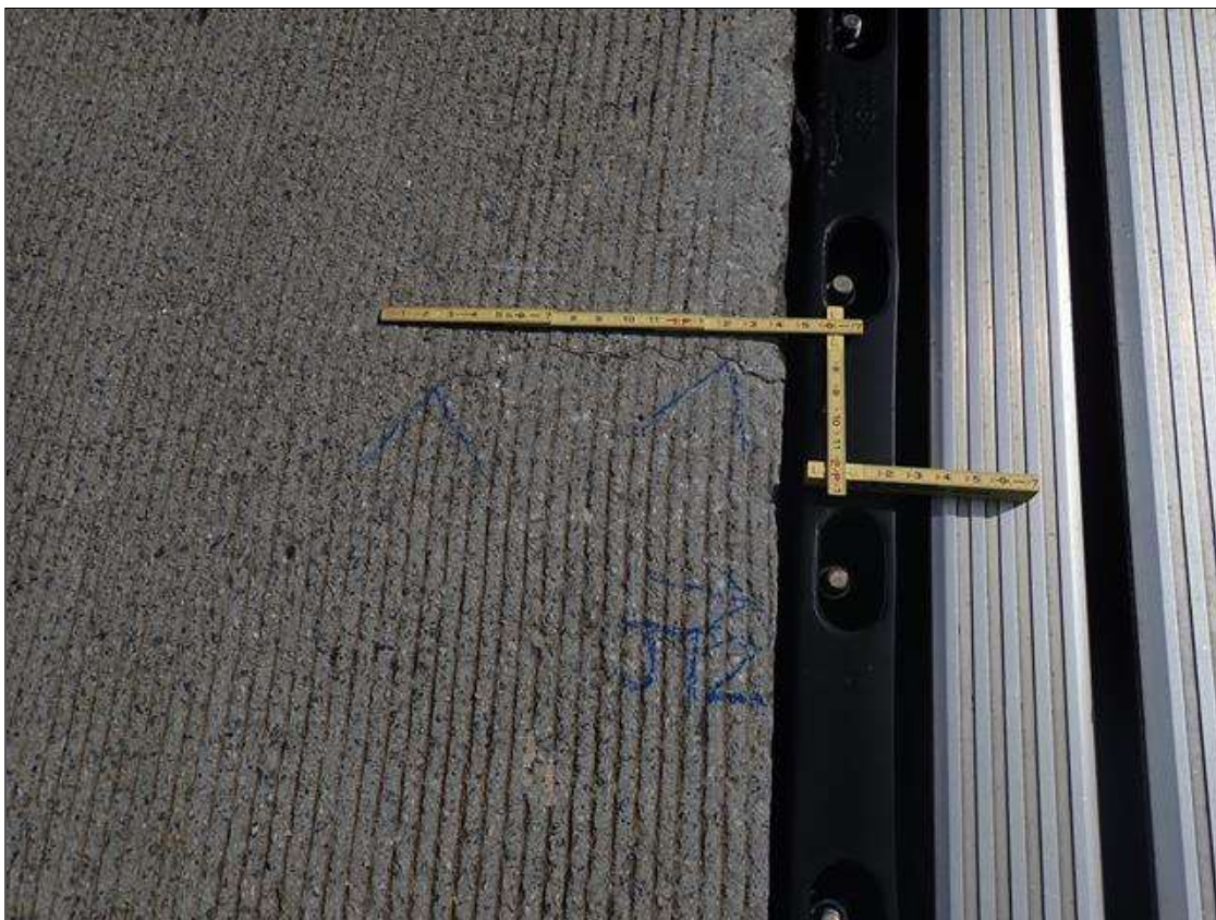
Span 2 Deck: left travel lane in right wheel path extending from joint 2, longitudinal crack [14in x 0.05in], extends down into joint
