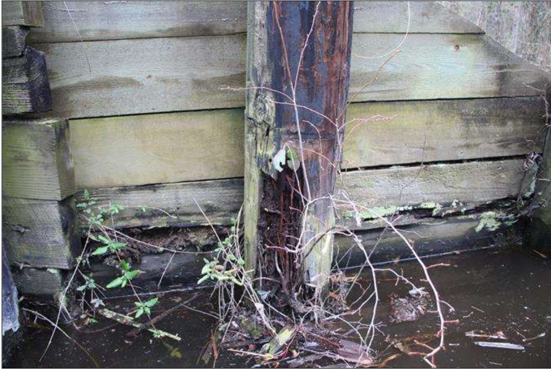
5 FT LONG X 9 IN HIGH X UP TO 3 IN DEEP AREA OF SEVERE DECAY WITH SOIL SPILLING THROUGH IN THE BOTTOM BULKHEAD BOARD. 2 FT HIGH X 3/4 IN DIAMETER X UP TO 3 IN DEEP AREA OF SEVERE DECAY AND TREE ROOTS IN THE FIRST SOLDIER PILE FROM SOUTH END OF THE ABUTMENT AT END BENT 1 (PAR).
