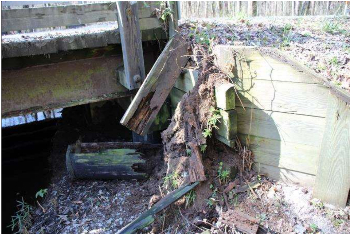
End Bent 1 Abutment/Backwall : SEVERE DETERIORATION OF SOLDIER PILE DUE TO DECAY AT NORTH END OF END BENT 1 ABUTMENT. 3 FT WIDE X 9 IN HIGH X 3 IN DEEP AREA OF BULKHEAD BOARD IS MISSING WITH SOIL SPILLING THROUGH. 10 IN WIDE X 6 IN HIGH X UP TO 3 IN DEEP AREA OF SECTION LOSS IN THE SECOND BULKHEAD BOARD IN BOTTOM AT NORTH END (PAR).
