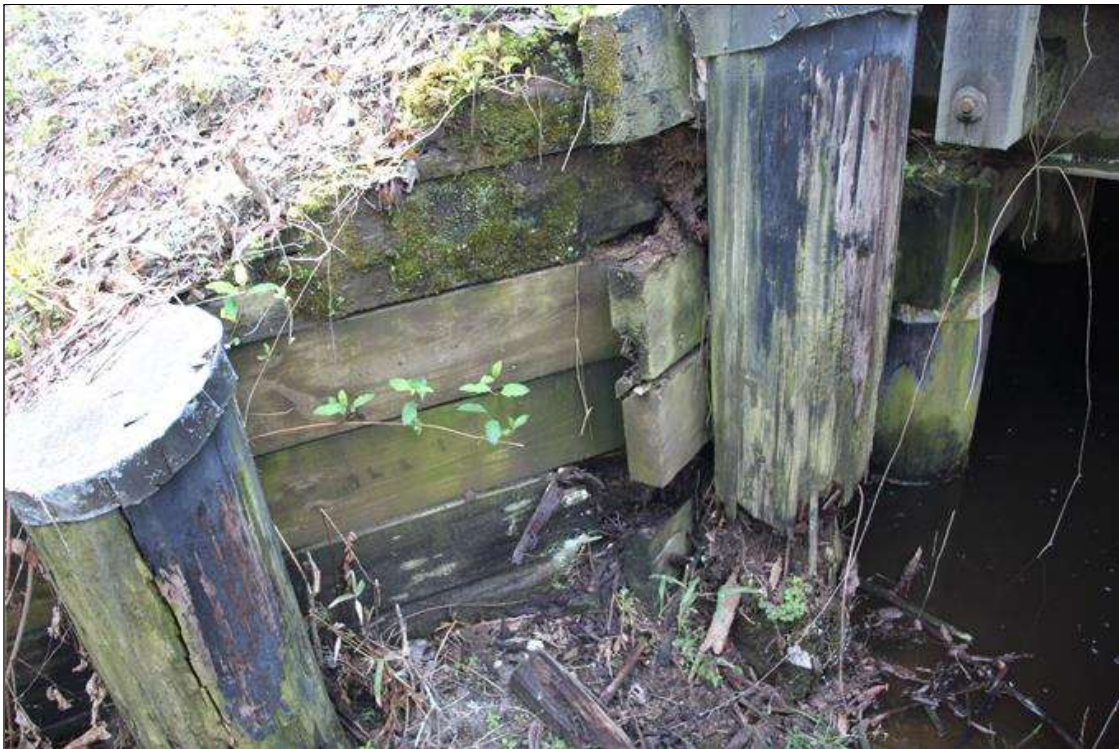
End Bent 2 Abutment/Backwall : UP TO 3 FT HIGH AREA OF SEVERE DECAY WITH UP TO 70% SECTION LOSS IN SOLDIER PILE AT NORTH END. 3 BULKHEAD BOARDS BEHIND THIS SOLDIER PILE EXHIBIT SEVERE DECAY UP TO 1 FT WIDE X 9 IN HIGH X 3 IN WIDE WITH SOIL SPILLING THROUGH (PAR).
