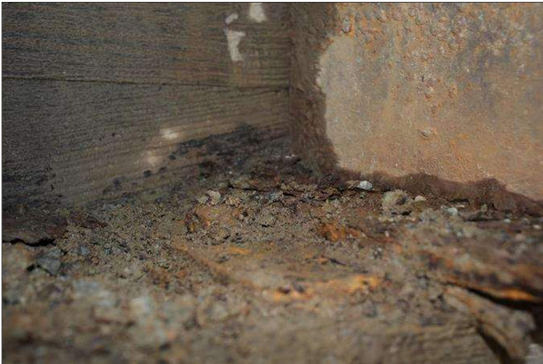
Span 1 Beam 3 Far Bearing: MODERATE TO HEAVY SURFACE CORROSION ON BEARING PLATE.
