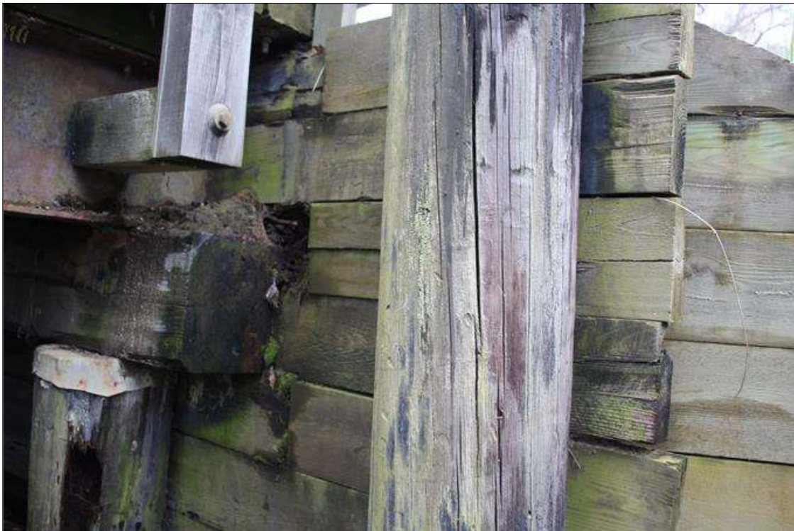
End Bent 2 Abutment/Backwall : UP TO 3/16 IN WIDE X 2 IN DEEP VERTICAL CHECKS IN SOUTHWEST FACE OF SOLDIER PILE AT SOUTH END.
