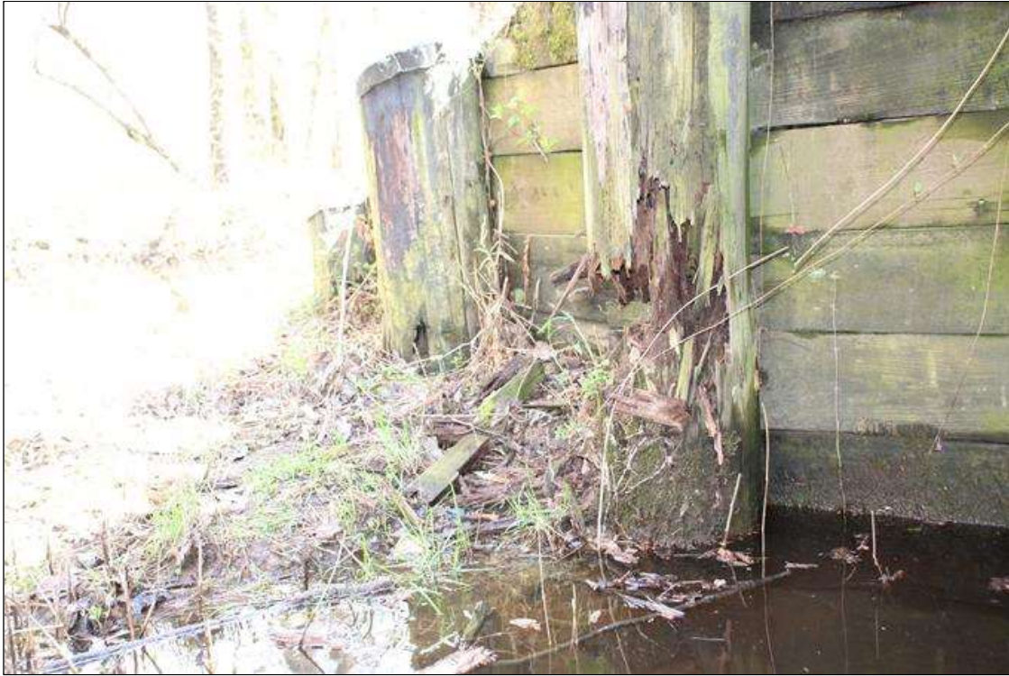
End Bent 2 Abutment/Backwall : UP TO 3 FT HIGH AREA OF SEVERE DECAY WITH UP TO 70% SECTION LOSS IN SOLDIER PILE AT NORTH END. 3 BULKHEAD BOARDS BEHIND THIS SOLDIER PILE EXHIBIT SEVERE DECAY UP TO 1 FT WIDE X 9 IN HIGH X 3 IN WIDE WITH SOIL SPILLING THROUGH (PAR).
