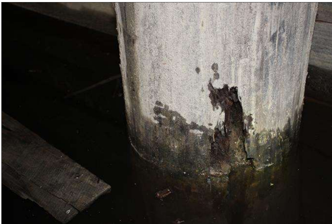
End Bent 2 Pile 3: 8 IN HIGH X 3 IN WIDE X 1 IN DEEP SECTION LOSS IN SOUTHWEST FACE, STARTING AT WATER LEVEL.
