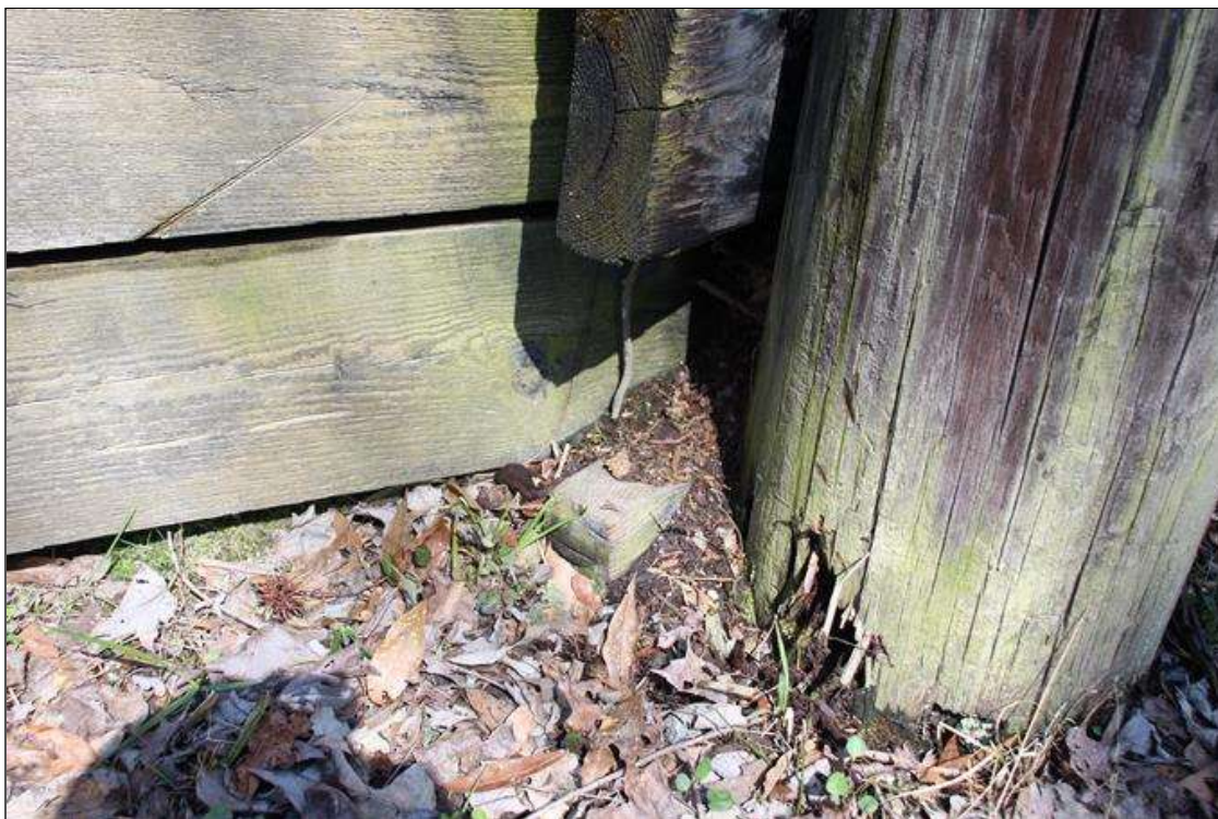
End Bent 1 Abutment/Backwall : 10 WIDE X 9 IN HIGH X 3IN DEEP AREA OF SECTION MISSING IN BOTTOM BULKHEAD BOARD AT SOUTH END.
