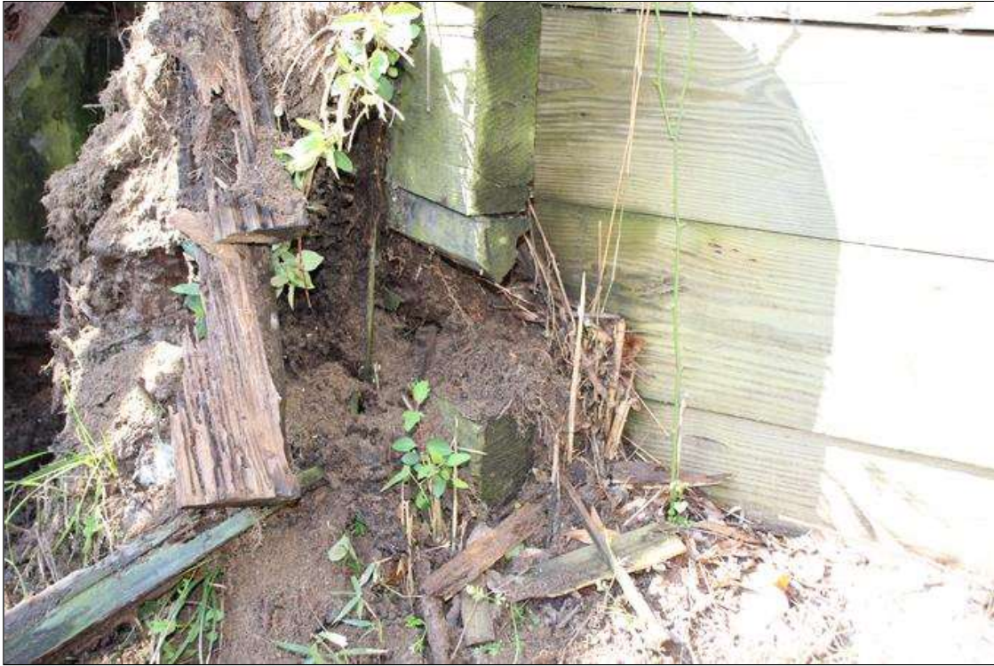
End Bent 1 Abutment/Backwall : SEVERE DETERIORATION OF SOLDIER PILE DUE TO DECAY AT NORTH END OF END BENT 1 ABUTMENT. 3 FT WIDE X 9 IN HIGH X 3 IN DEEP AREA OF BULKHEAD BOARD IS MISSING WITH SOIL SPILLING THROUGH. 10 IN WIDE X 6 IN HIGH X UP TO 3 IN DEEP AREA OF SECTION LOSS IN THE SECOND BULKHEAD BOARD IN BOTTOM AT NORTH END (PAR).
