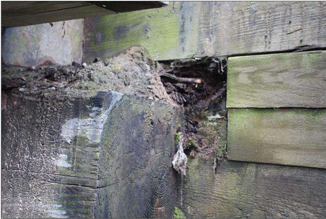
End Bent 2 Abutment/Backwall : UP TO 1 FT WIDE X 8 IN HIGH X 3 IN DEEP AREA OF DECAY AND SECTION LOSS WITH SOIL SPILLING THROUGH BEHIND THE CAP AT SOUTH END OF END BENT 2 (PAR).
