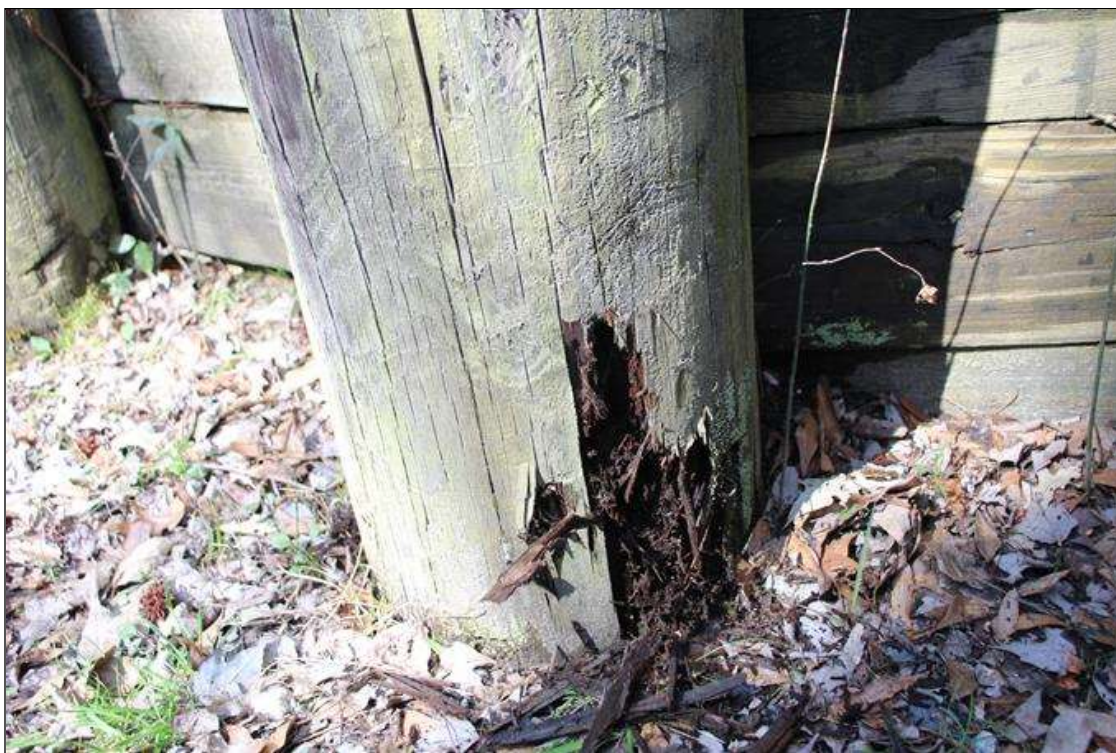
End Bent 1 Abutment/Backwall : UP TO 8 IN HIGH X FULL DIAMETER OF THE BOTTOM SOLDIER PILE HAS MODERATE DECAY AT THE GROUND SURFACE.
