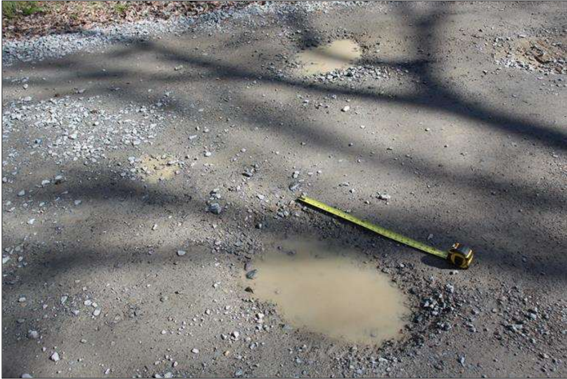
TWO (2) POTHOLES UP TO 2.5 FT X 2 FT LONG X 3 IN DEEP IN WEST APPROACH PAVEMENT.
