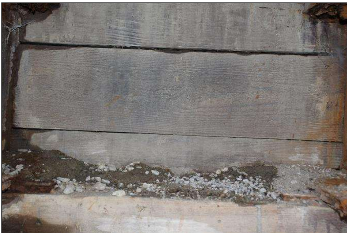
End Bent 1 Cap 1: MODERATE TO HEAVY DIRT AND DEBRIS ON TOP OF THE CAP IN BAYS 2, 4, AND 6. PHOTO SHOWS DEBRIS IN BAY 4.
