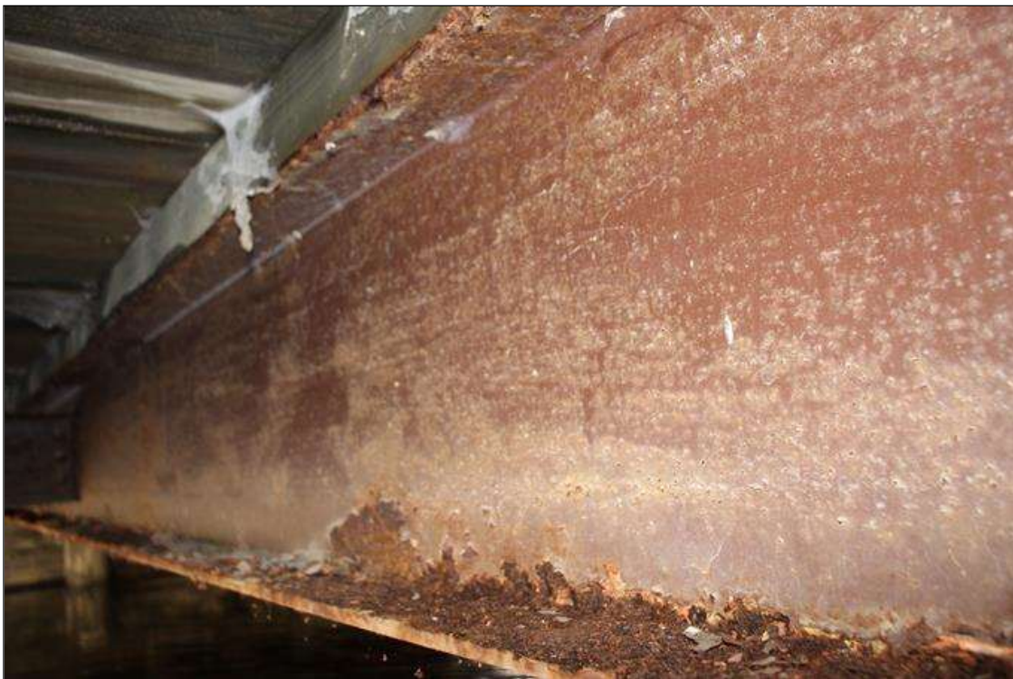
Span 1 Beam 2: MODERATE SURFACE CORROSION ON EDGES OF TOP FLANGES THROUGHOUT AND IN AREAS ON THE BOTTOM FLANGE.
