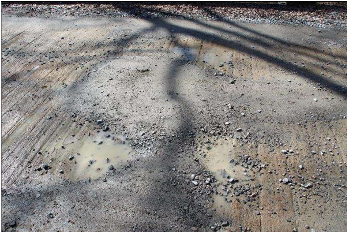
Span 1 Deck: 4 FT LONG X 4 FT WIDE SOUND CONCRETE PATCH AT THE BEGINNING OF THE BRIDGE.
