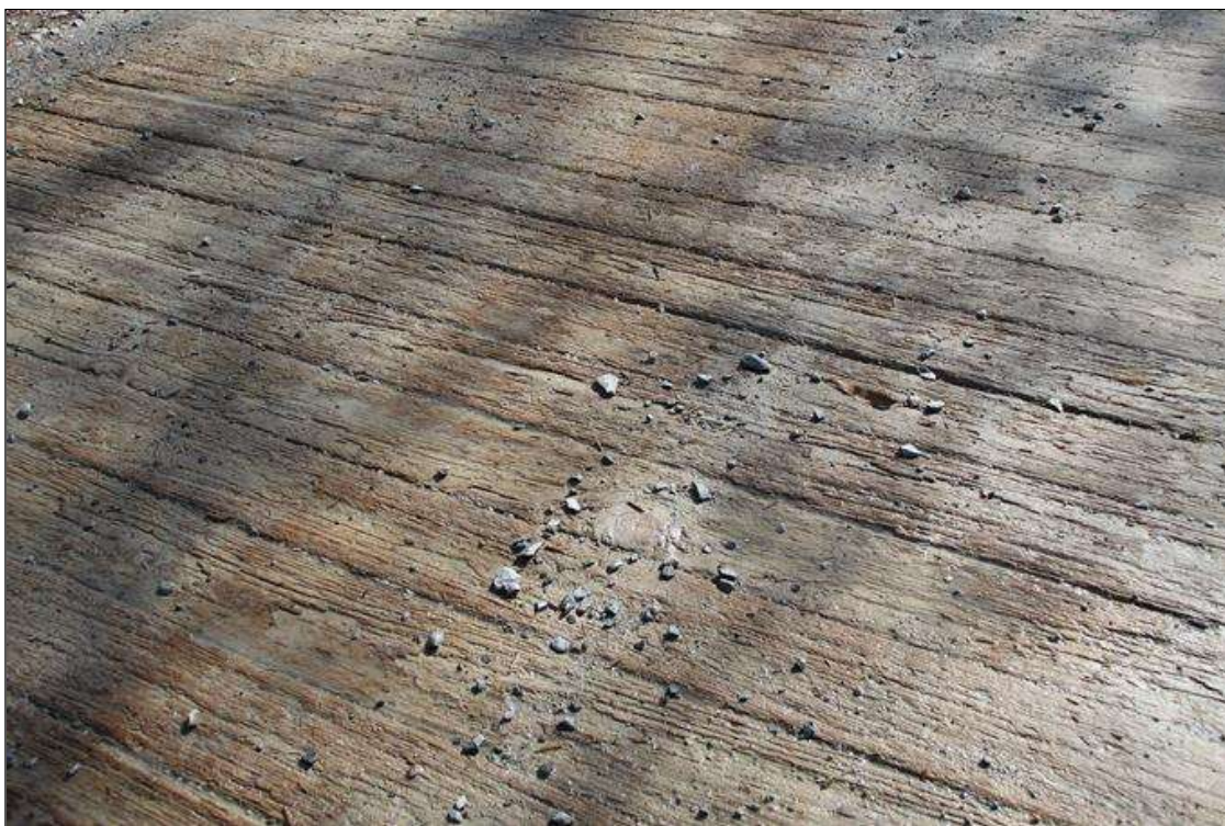
Span 1 Deck: MINOR TO MODERATE ABRASION WITH WATER PONDING ON EXPOSED TIMBER BOARDS FOR UP TO 70% OF DECK AREA.
