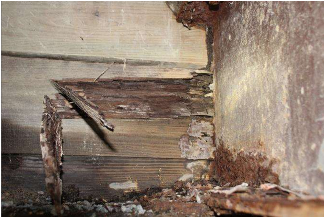
End Bent 2 Abutment/Backwall : 3 FT WIDE X 1 FT HIGH X 3 IN DEEP AREA OF SEVERE DECAY IN THE BACKWALL BULKHEAD BOARDS BEHIND BEAM 5 AND IN BAY 5 WITH SOIL SPILLING THROUGH (PAR).
