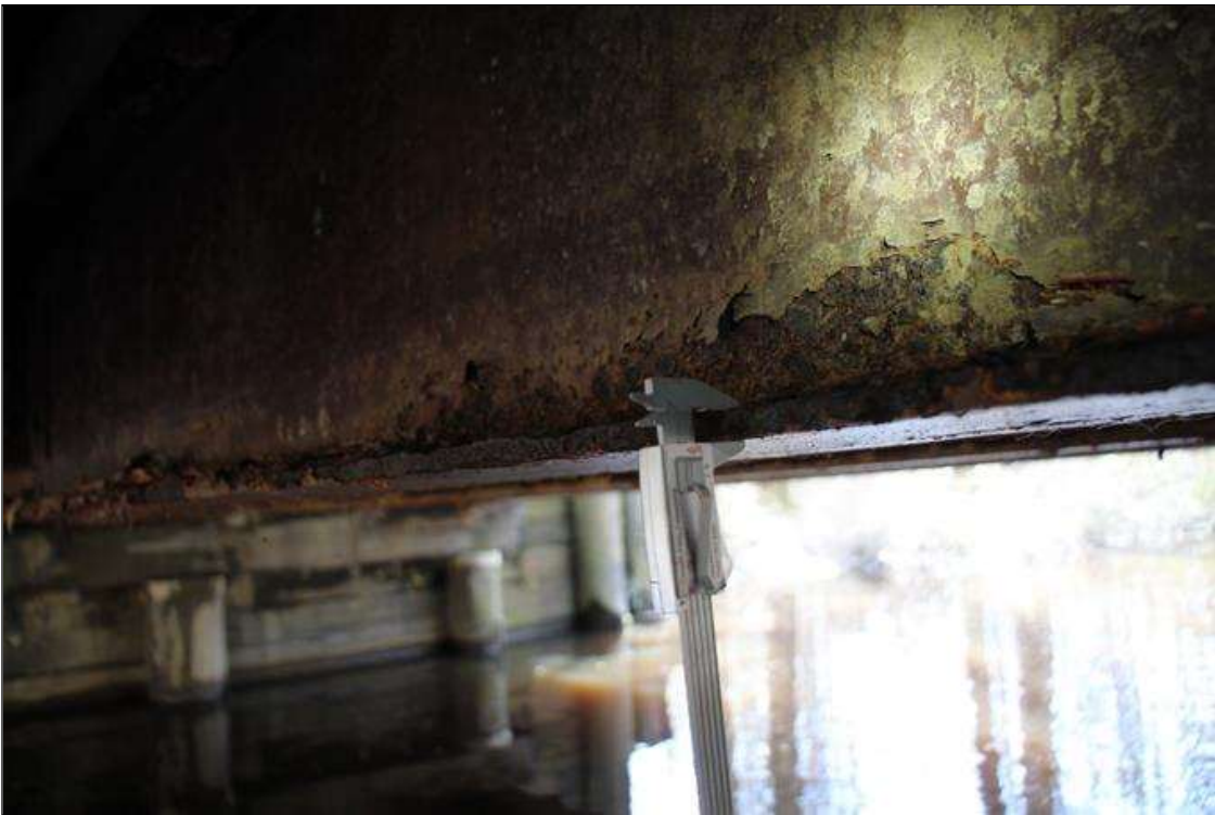
Span 1 Beam 4: HEAVY SURFACE CORROSION FOR FULL FLANGE WIDTH X 18.5 FT LONG IN BOTTOM FLANGE, STARTING AT 7.5 FT FROM BEAM END AT END BENT 1 . UP TO 0.36 IN SECTION REMANING (PAR).
