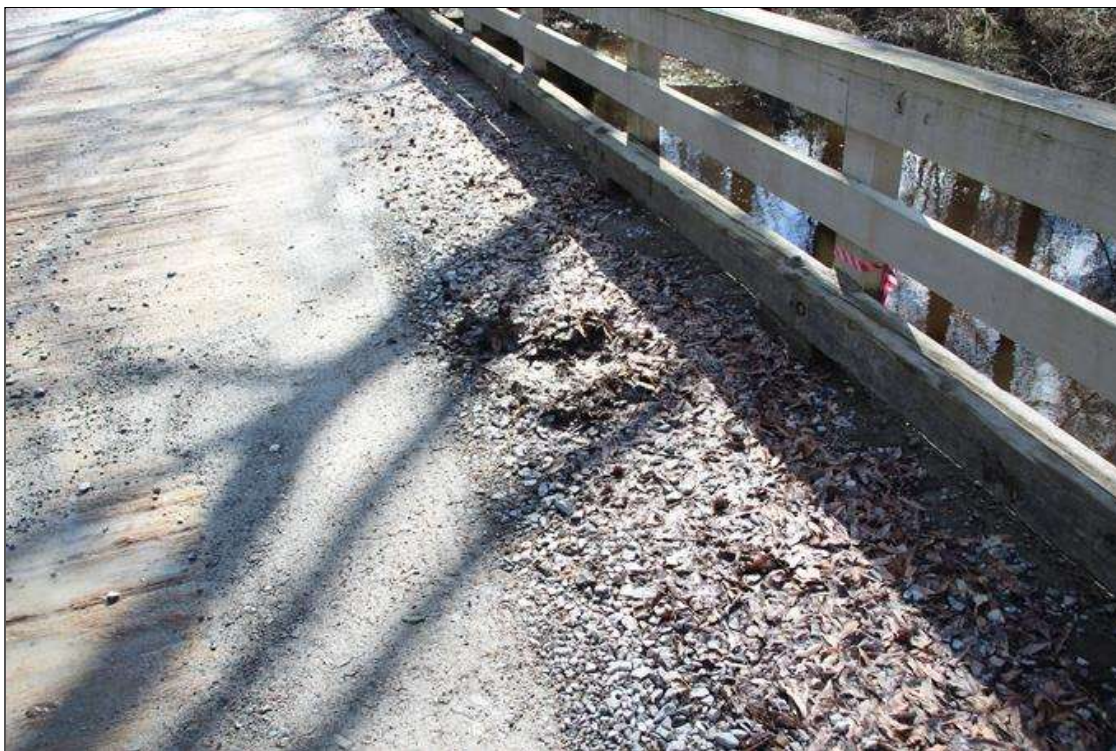
Span 1 Deck: LOOSE AGGREGATE FOR 3 FT WIDE X FULL SPAN LENGTH ALONG BOTH BRIDGE RAILS.
