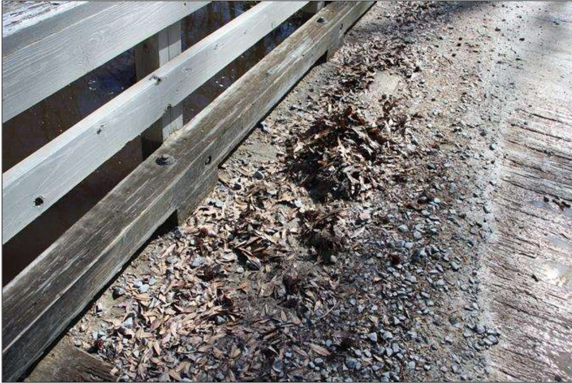
MODERATE TO HEAVY DEBRIS AND DRY LEAVES ACCUMULATED ALONG BOTH BRIDGE RAILS.
