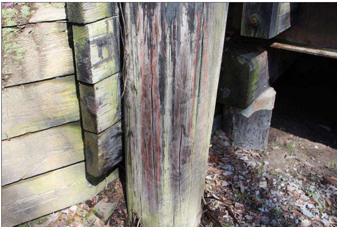
End Bent 1 Abutment/Backwall : 3/16 IN WIDE X 1 IN DEEP VERTICAL CHECKS FOR FULL HEIGHT IN SOUTH FACE.
