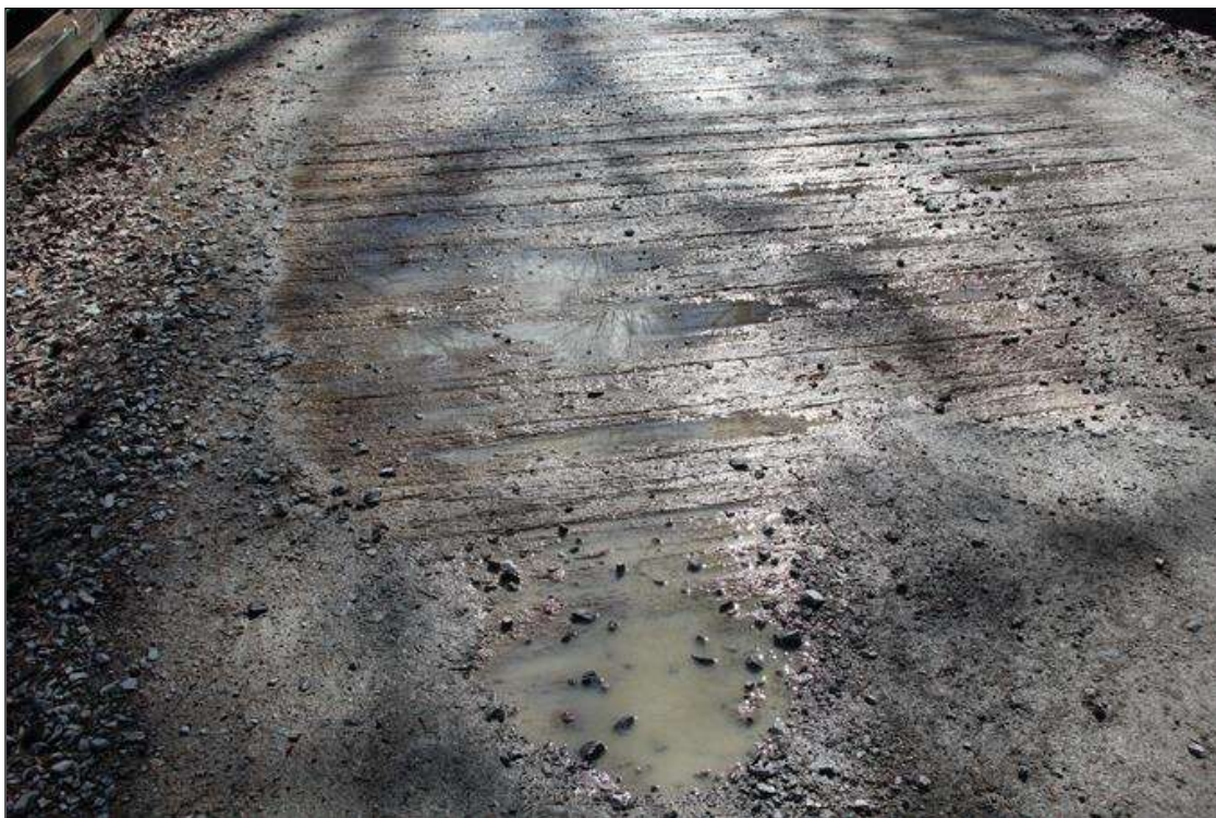
Span 1 Deck: MINOR TO MODERATE ABRASION WITH WATER PONDING ON EXPOSED TIMBER BOARDS FOR UP TO 70% OF DECK AREA.
