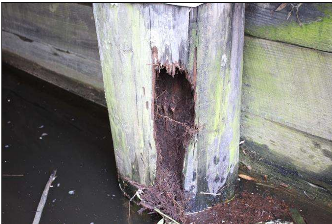
End Bent 2 Pile 4: 20 IN HIGH X 5 IN WIDE X UP TO 3 IN DEEP AREA OF SECTION LOSS DUE TO DECAY STARTING AT WATER LEVEL IN SOUTHWEST CORNER (PAR).
