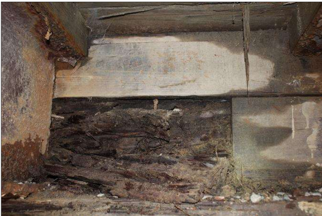
End Bent 2 Abutment/Backwall : 3 FT WIDE X 1 FT HIGH X 3 IN DEEP AREA OF SEVERE DECAY IN THE BACKWALL BULKHEAD BOARDS BEHIND BEAM 5 AND IN BAY 5 WITH SOIL SPILLING THROUGH (PAR).
