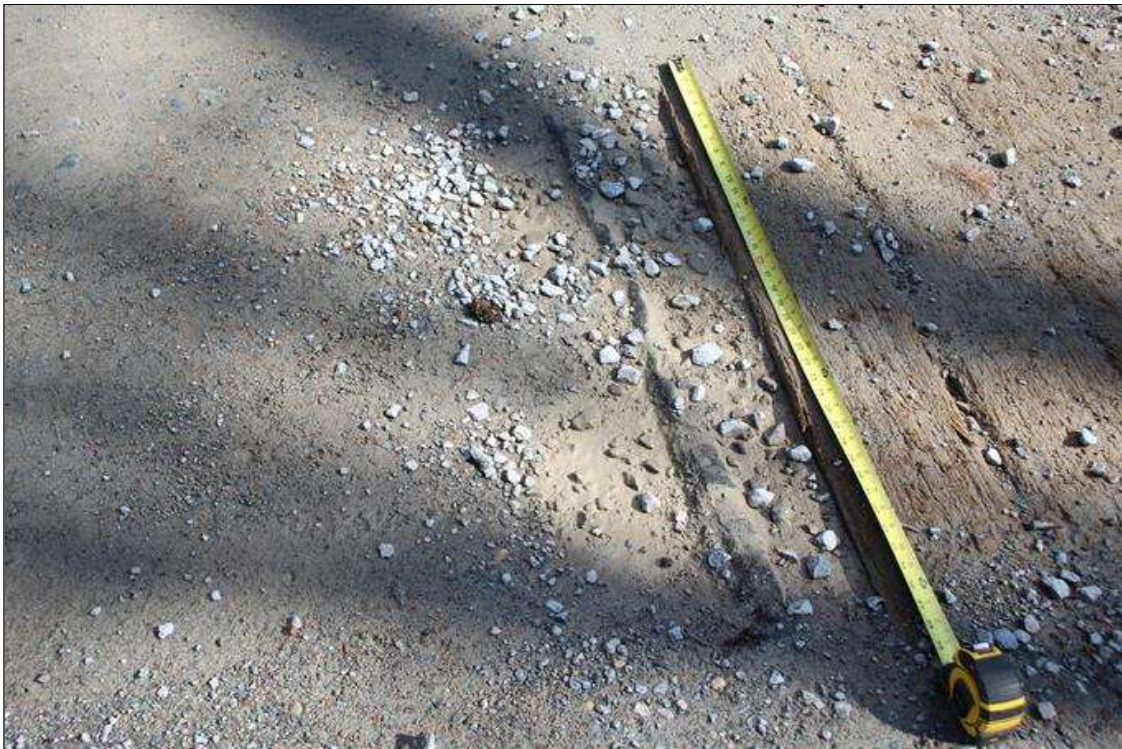
3 FT WIDE X 1.5 FT LONG X UP TO 2 IN DEEP POTHOLE IN RIGHT LANE AT DECK JOINT IN WEST APPROACH PAVEMENT.
