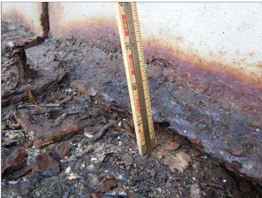
Span 1 Beam 1: SECTION LOSS BENT 1 BOTTOM FLANGE 1/8 IN REMAINING 4 FOOT LONG, WEB 5/16 IN REMAINING 3 IN HIGH PRIORITY MAINTENANCE ISSUED
