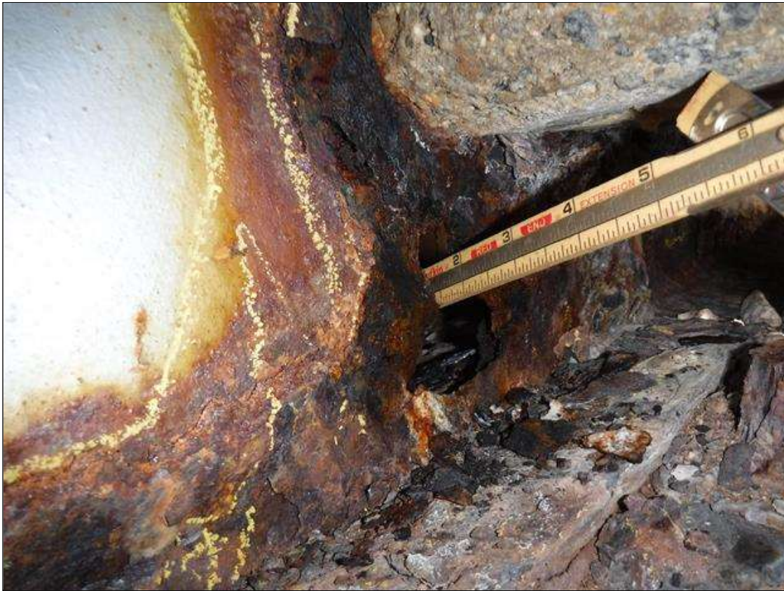
Span 4 Beam 9: SECTION LOSS WEB BENT 4 - HOLE 3 IN DIAMETER , SECTION LOSS 100 % BOTTOM FLANGE 1 1/2 IN WIDE X 2 FOOT LONG PRIORITY MAINTENANCE ISSUED
