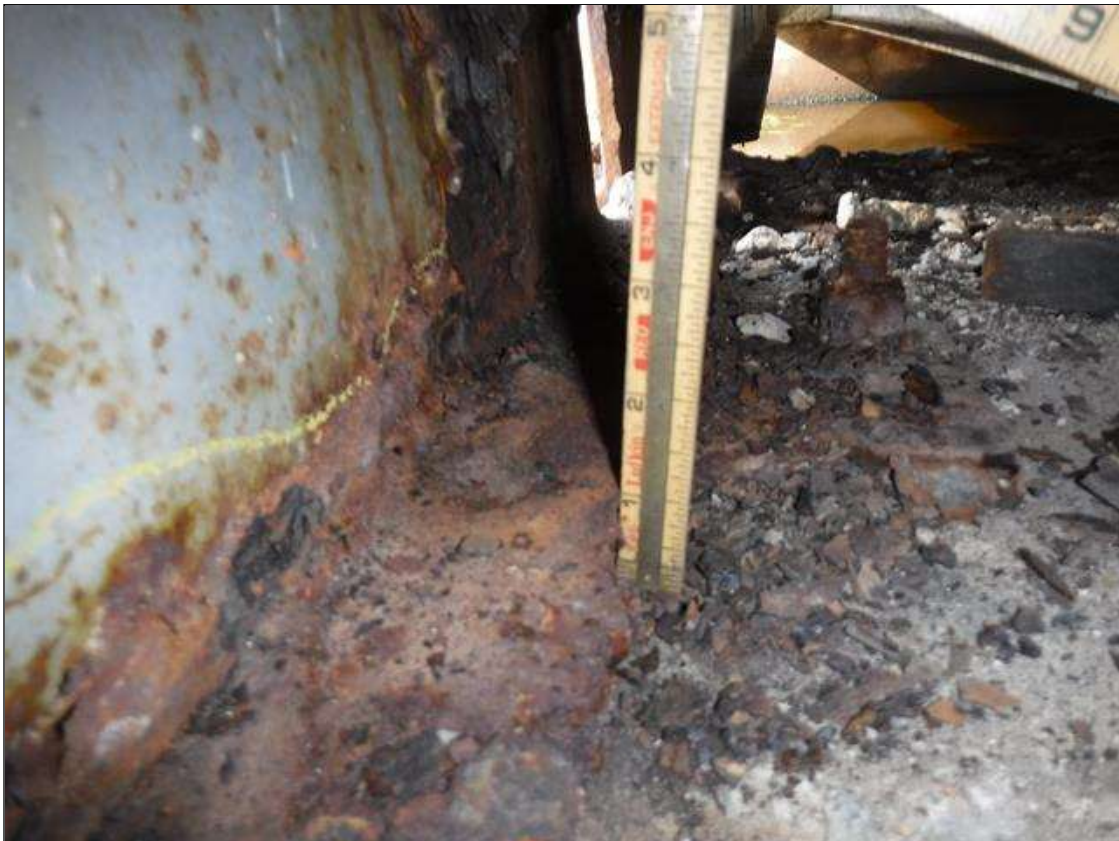
Span 2 Beam 10: SECTION LOSS 1/8 IN REMAINING 2 FOOT LONG BOTTOM FLANGE BENT 1 PRIORITY MAINTENANCE ISSUED
