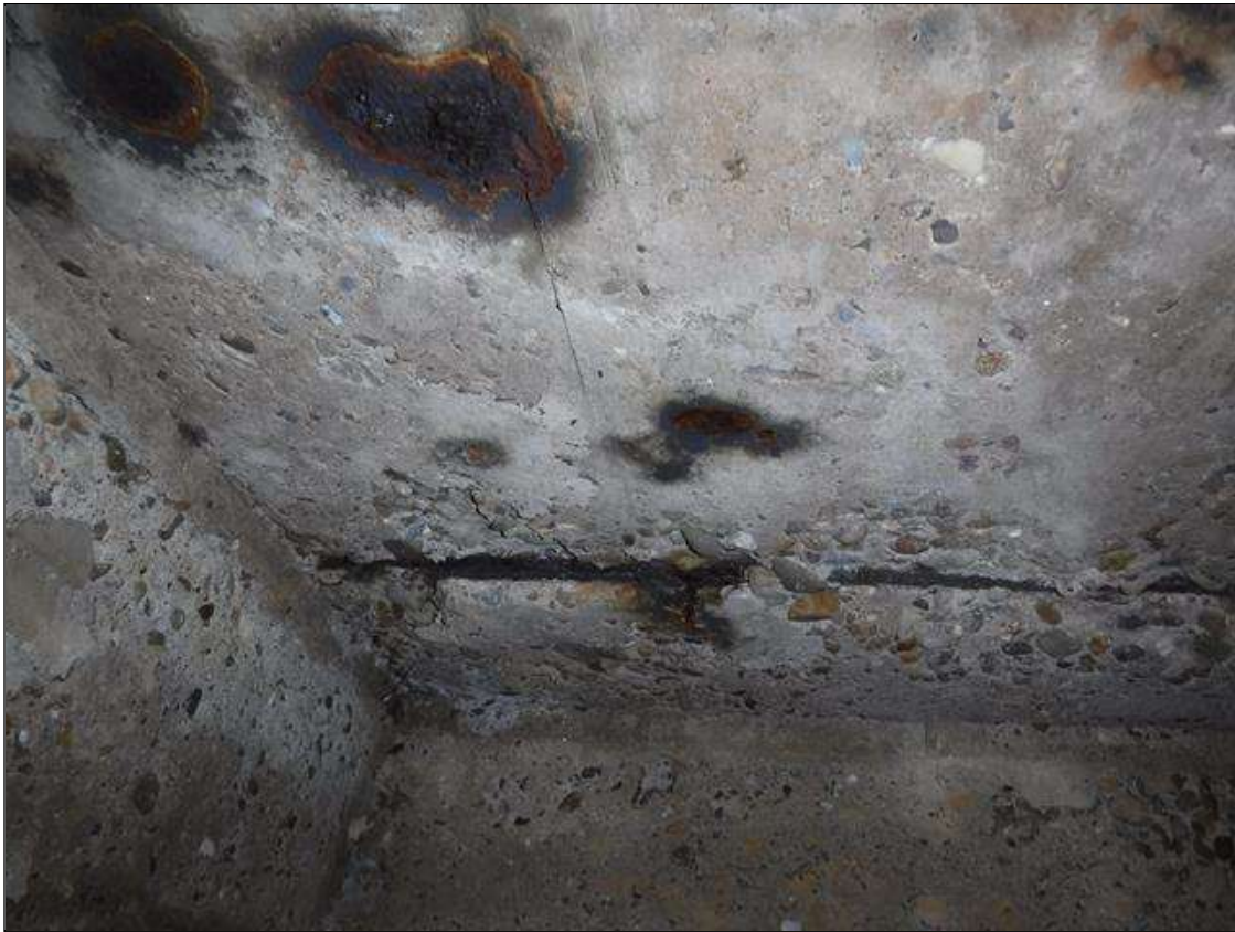
Span 5 Deck: SURFACE SPALLS WITH EXPOSED STEEL UNDER BAY 3
