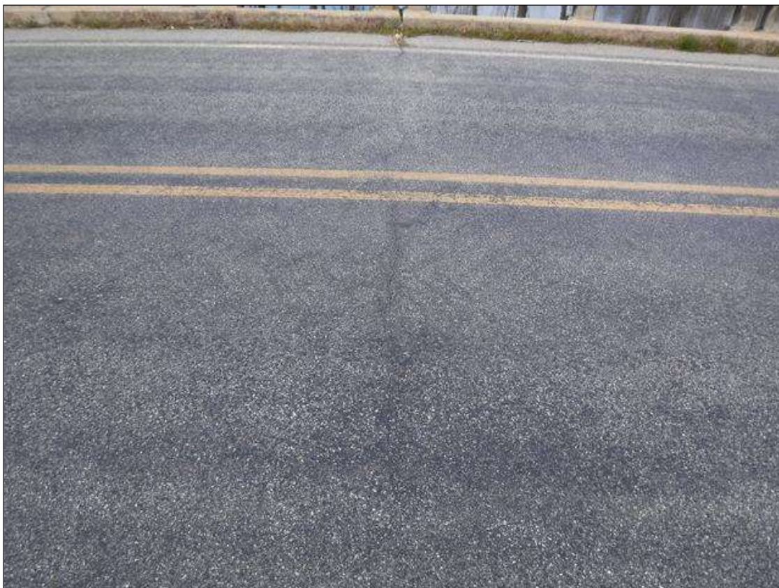
Span 1 Wearing Surface: TRANSVERSE CRACKING OVER BENT 1 END BENT 1 SIMILAR
