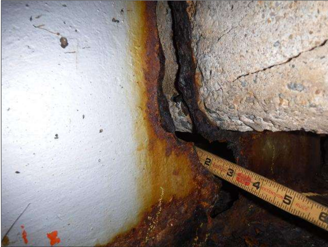
Span 3 Beam 9: SECTION LOSS BENT 3 WEB - HOLE 3 IN X 10 IN HIGH , SECTION LOSS BOTTOM FLANGE 100 % 1 IN WIDE X 16 IN LONG PRIORITY MAINTENANCE ISSUED
