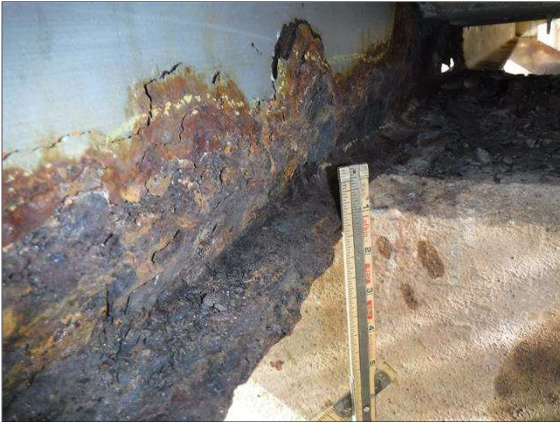
Span 2 Beam 9: SECTION LOSS BOTTOM FLANGE AT BENT 1 -100 % 1 IN WIDE X 4 FOOT LONG , WEB 5/16 IN REMAINING 3 IN HIGH PRIORITY MAINTENANCE ISSUED
