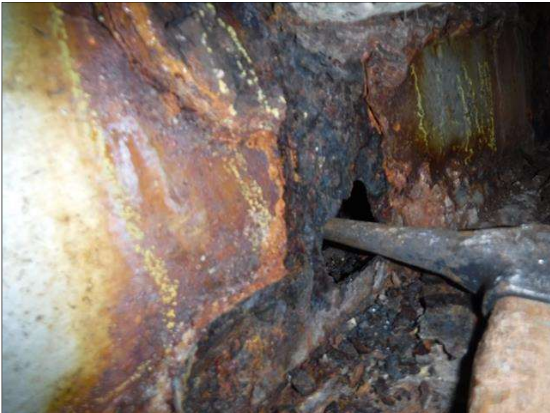
Span 4 Beam 2: SECTION LOSS BENT 3 BOTTOM FLANGE 1.5" DIAMETER HOLE IN WEB 100 % 1 IN WIDE X 18 IN LONG , 5/16 IN REMAINING WEB 3 IN HIGH PRIORITY MAINTENANCE ISSUED
