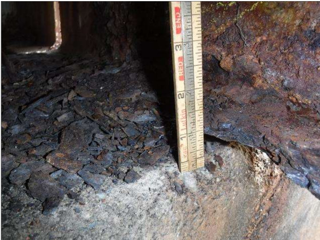
Span 4 Beam 10: SECTION LOSS 100 % IN BOTTOM FLANGE BENT 4 1 IN WIDE X 16 IN LONG , 5/16 IN REMAINING WEB 4 IN HIGH PRIORITY MAINTENANCE ISSUED
