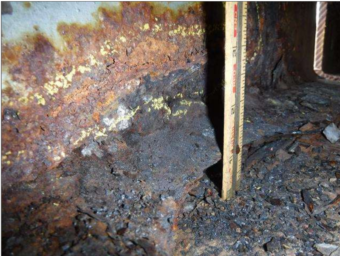
Span 5 Beam 10: 100 % SECTION LOSS BOTTOM FLANGE BENT 4 - 1.5 IN WIDE X 18 IN LONG , 5/16 IN REMAINING 2 IN HIGH WEB
