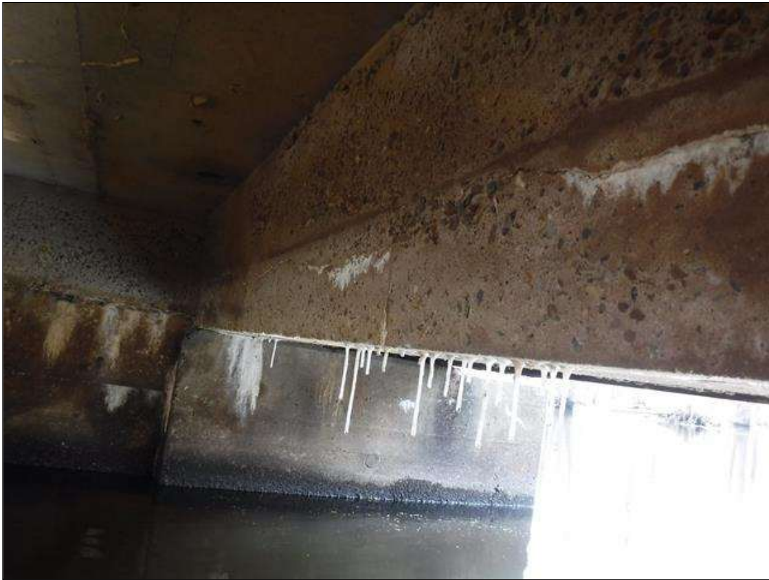
Span 2 Beam 8: CRACKING WITH EFFLO
