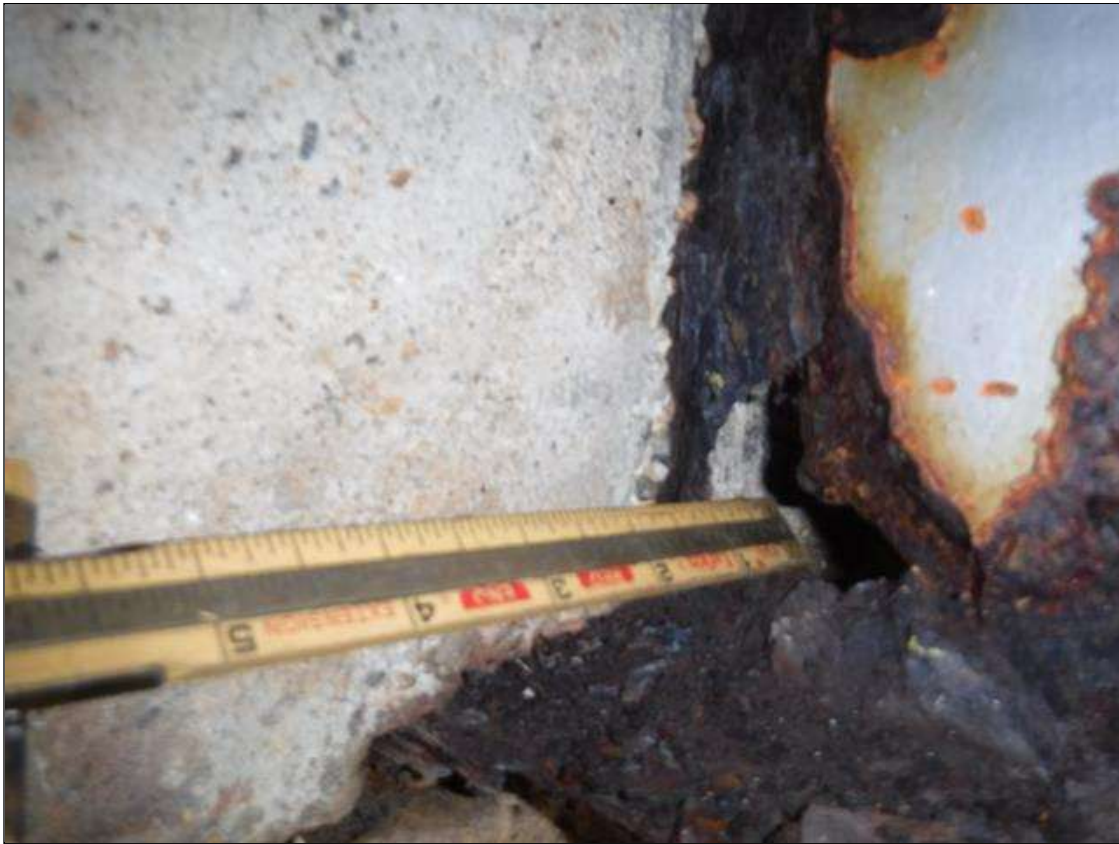
Span 5 Beam 2: SECTION LOSS ABUTMENT 2 WEB - HOLE 1.5 IN DIAMETER , 100 % SECTION LOSS BOTTOM FLANGE 1/2 IN WIDE X 3 IN LONG PRIORITY MAINTENANCE ISSUED
