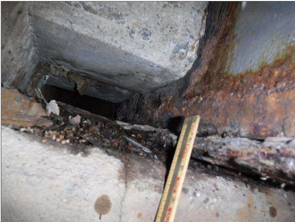
Span 5 Beam 2: SECTION LOSS BOTTOM FLANGE AT BENT 4 - 1/8 IN REMAINING 3 FOOT LONG , 5/16 IN REMAINING WEB 2 IN HIGH PRIORITY MAINTENANCE ISSUED
