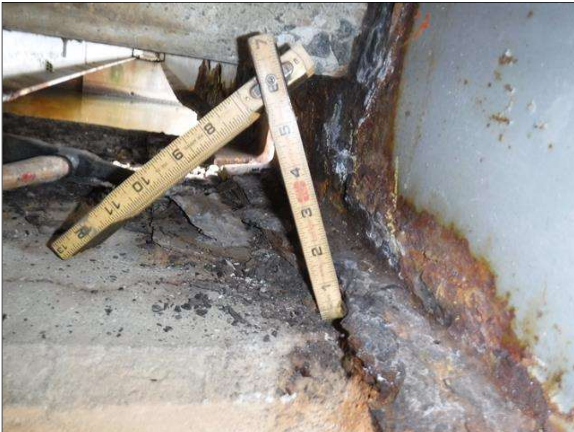
Span 3 Beam 10: SECTION LOSS 100 % 1 IN WIDE X 18 IN LONG AT BENT 3 BOTTOM FLANGE, 1/4 IN REMAINING WEB 4 IN HIGH PRIORITY MAINTENANCE ISSUED
