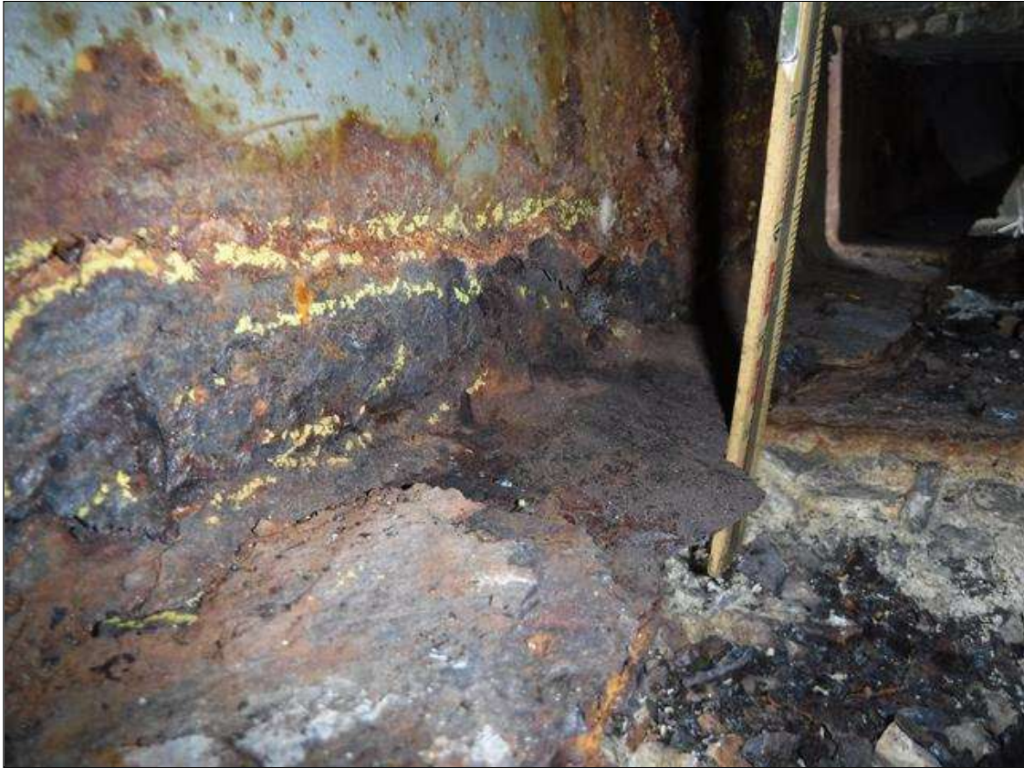
Span 2 Beam 1: SECTION LOSS BOTTOM FLANGE AT BENT 2 -100 % 1 IN WIDE X 2 FOOT LONG , WEB 5/16 IN REMAINING 3 IN HIGH PRIORITY MAINTENANCE ISSUED
