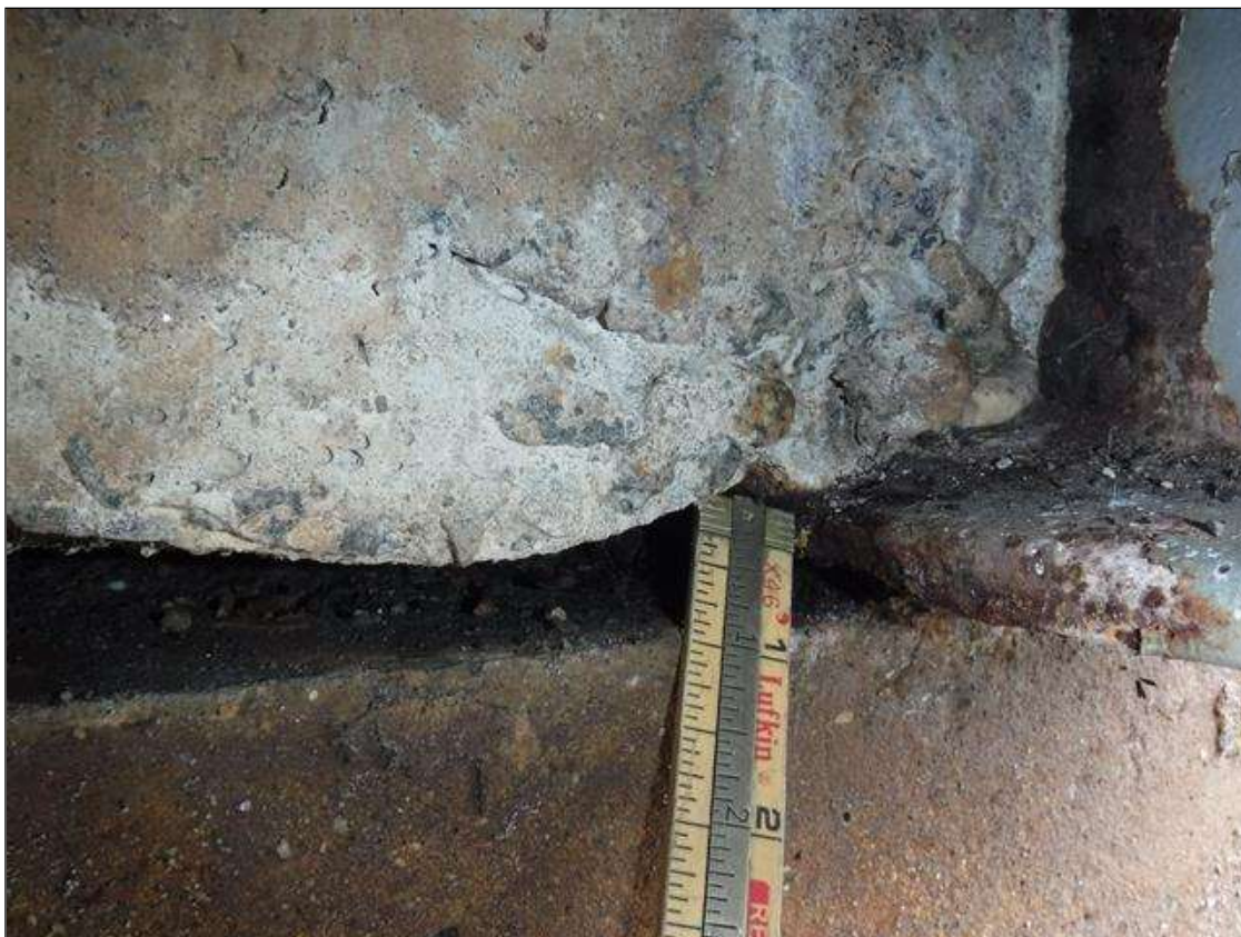
Span 1 Beam 1: SECTION LOSS BOTTOM FLANGE ABUTMENT 1 - 1/4 IN REMAINING 2 IN LONG PRIORITY MAINTENANCE ISSUED
