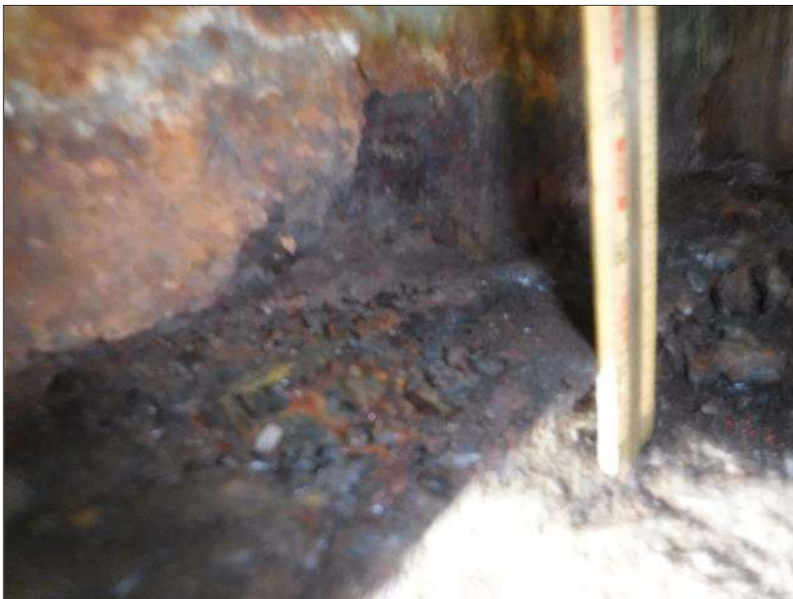
Span 4 Beam 1: SECTION LOSS BENT 4 BOTTOM FLANGE 100 % 1/2 IN WIDE X 18 IN LONG PRIORITY MAINTENANCE ISSUED
