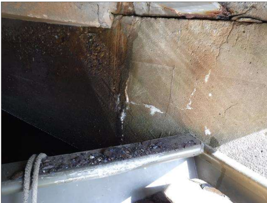
End Bent 2 Abutment/Backwall : CRACKING IN FACE OF CAP UNDER BEAM 9
