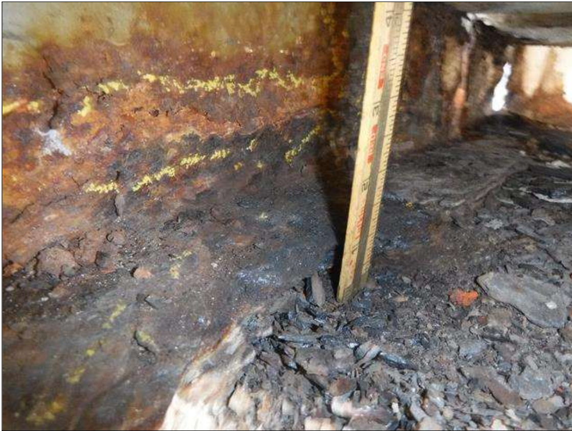
Span 5 Beam 9: 1 IN HOLE 4 IN HIGH END WEB BENT 4 , 100 % SECTION LOSS BOTTOM FLANGE 1 IN WIDE X 18 IN LONG PRIORITY MAINTENANCE ISSUED
