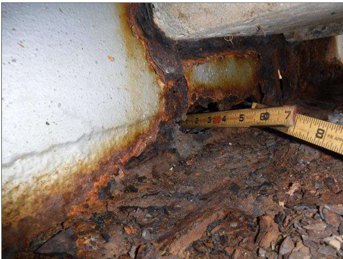
Span 1 Beam 9: SECTION LOSS WEB BENT 1 - HOLE 2 IN HIGH X 8 IN LONG , BOTTOM FLANGE 100 % SECTION LOSS 1 N WIDE X 1 FOOT LONG PRIORITY MAINTENANCE ISSUED
