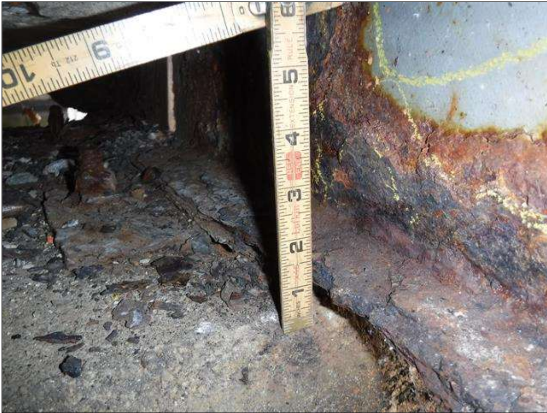
Span 4 Beam 1: SECTION LOSS BENT 3 BOTTOM FLANGE 100 % 1 IN WIDE X 2 FOOT LONG , WEB 5/16 IN REMAINING 4 IN HIGH PRIORITY MAINTENANCE ISSUED
