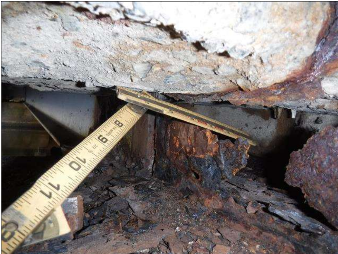
Span 3 Beam 2: SECTION LOSS WEB BENT 3 - HOLE 4 IN X 12 IN , SECTION LOSS BOTTOM FLANGE 100 % 1 IN WIDE X 12 IN LONG PRIORITY MAINTENANCE ISSUED
