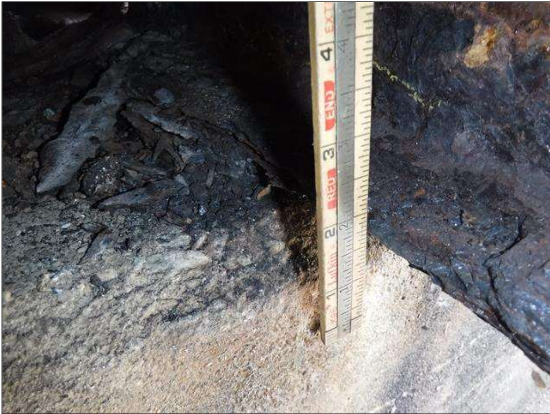
Span 5 Beam 1: SECTION LOSS 100 % IN BOTTOM FLANGE BENT 4 - 1/2 IN WIDE X 4 FOOT LONG, 5/16 IN REMAINING WEB 3 IN HIGH PRIORITY MAINTENANCE ISSUED
