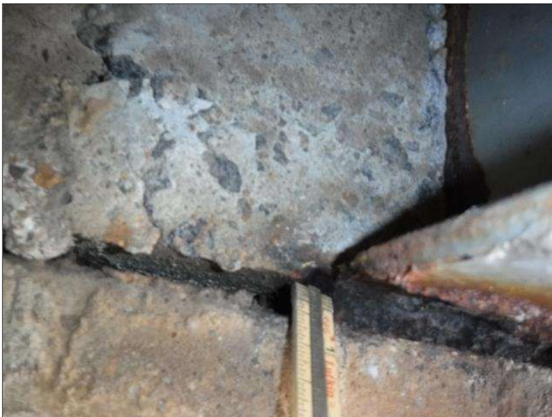
Span 1 Beam 2: SECTION LOSS BOTTOM FLANGE ABUTMENT 1 2 IN LONG 1/4 IN REMAINING PRIORITY MAINTENANCE ISSUED
