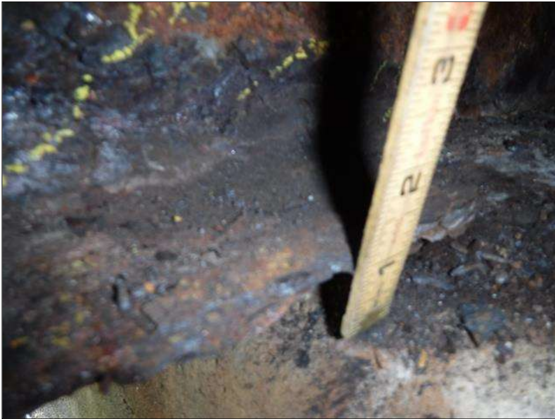
Span 4 Beam 9: SECTION LOSS 100 % BOTTOM FLANGE BENT 3 -1 IN WIDE X 2 FOOT LONG , 5/16 IN REMAINING WEB 2 IN HIGH PRIORITY MAINTENANCE ISSUED
