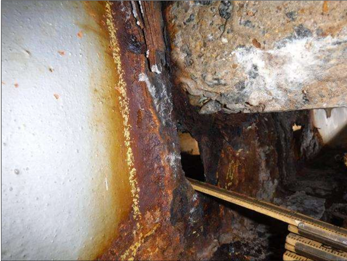
Span 2 Beam 9: SECTION LOSS BEAM BENT 2 - 2" DIAMETER HOLE 100 % 1 IN WIDE X 3 FOOT LONG , WEB 5/16 IN REMAINING 3 IN HIGH PRIORITY MAINTENANCE ISSUED
