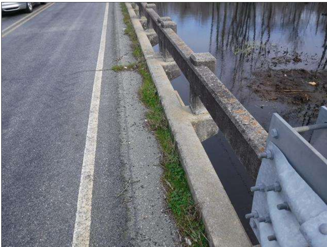
DEBRIS ALONG GUARDRAIL
