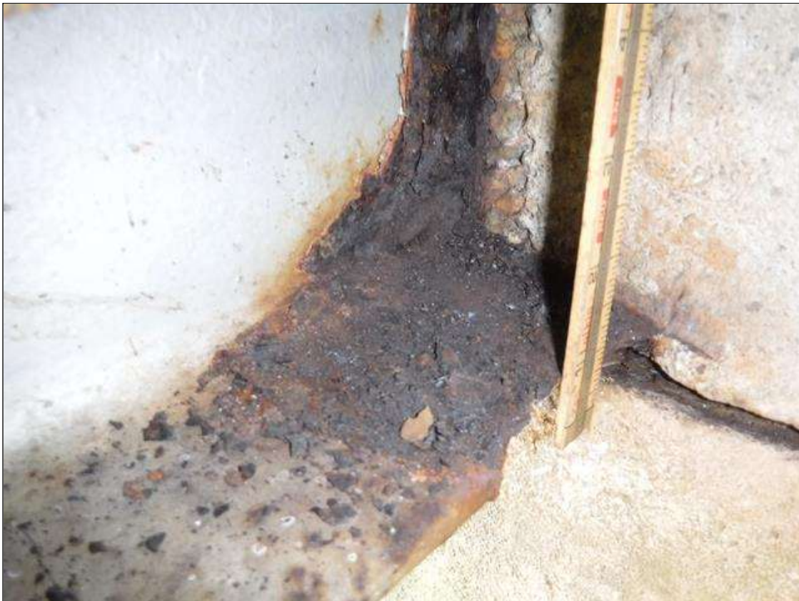
Span 5 Beam 1: SECTION LOSS IN BOTTOM FLANGE AT ABUTMENT 2 - 100 % 3/4 IN WIDE X 2 IN LONG PRIORITY MAINTENANCE ISSUED
