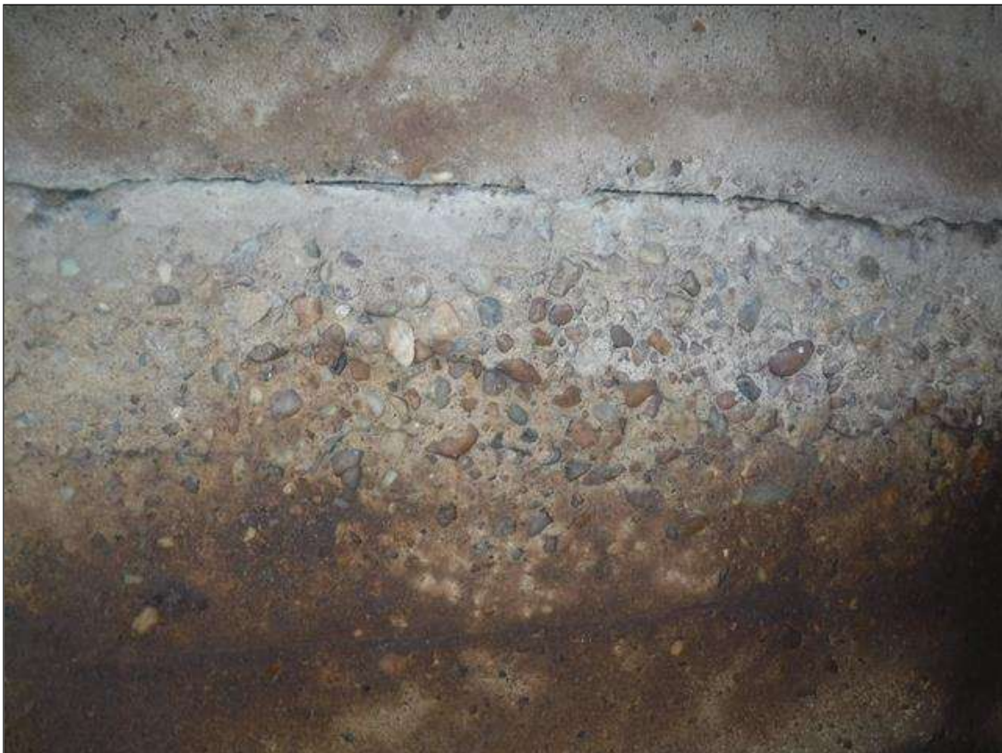
End Bent 2 Abutment/Backwall : ABRASION
