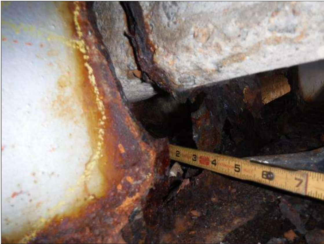
Span 2 Beam 2: SECTION LOSS BENT 1 WEB - HOLE 6 IN WIDE X 6 IN HIGH REST OF AREA 1/16 IN REMAINING, SECTION LOSS BEAM 1/8 IN REMAINING 1 FOOT LONG PRIORITY MAINTENANCE ISSUED
