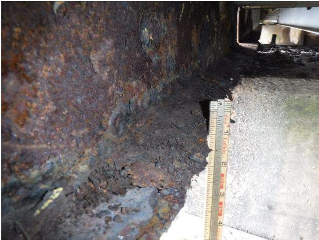
Span 3 Beam 10: SECTION LOSS EDGE BOTTOM FLANGE BENT 2 100 % 1/2 IN WIDE X 4 FOOT LONG , 5/16 IN REMAINING WEB 5 IN HIGH PRIORITY MAINTENANCE ISSUED
