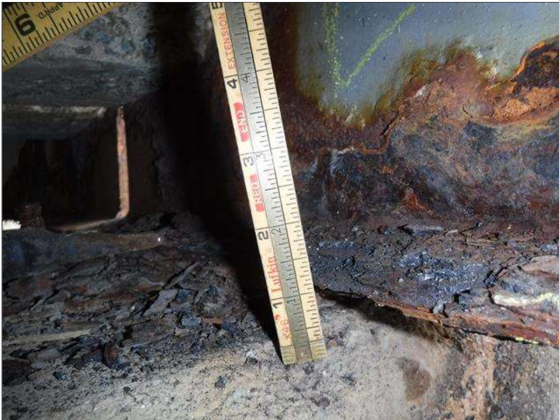
Span 2 Beam 10: SECTION LOSS BOTTOM FLANGE BENT 2 - 1/8 IN REMAINING 4 FOOT LONG , WEB 5/16 IN REMAINING 3 IN HIGH X 4 FOOT LONG PRIORITY MAINTENANCE ISSUED
