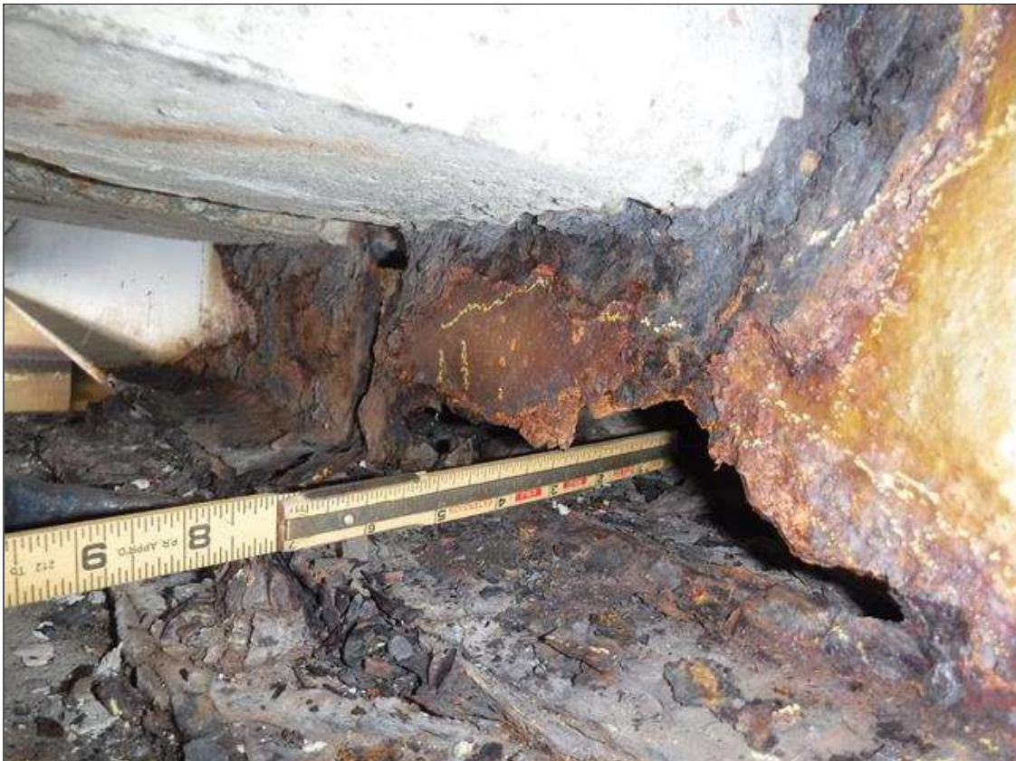
Span 2 Beam 2: SECTION LOSS WEB BENT 2 - HOLE 2 IN X 8 IN LONG BOTTOM FLANGE 100 % SECTION LOSS 1 IN WIDE X 16 IN LONG PRIORITY MAINTENANCE ISSUED
