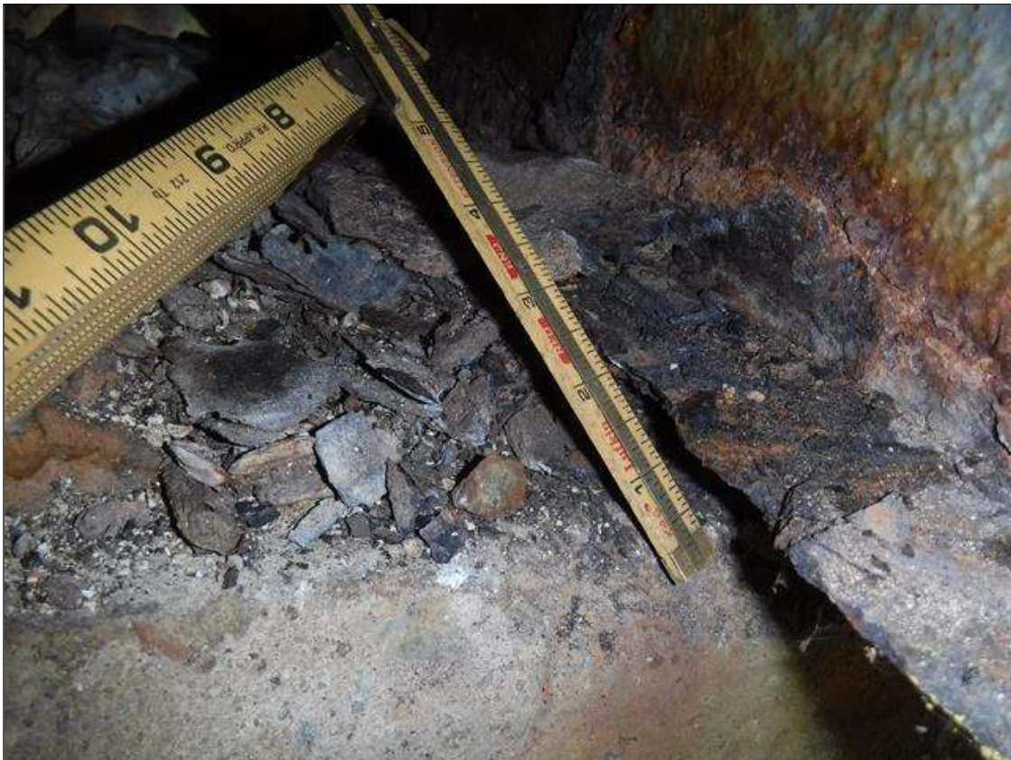
Span 3 Beam 2: SECTION LOSS BENT 2 BOTTOM FLANGE 1/8 IN REMAINING 2 FOOT PRIORITY MAINTENANCE ISSUED
