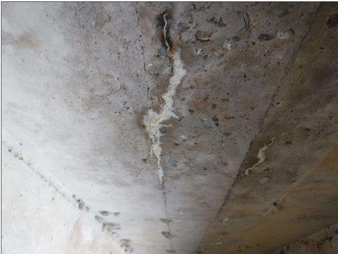
Span 2 Deck: EFFLO LEAKAGE IN BOTTOM OF DECK BAY 5
