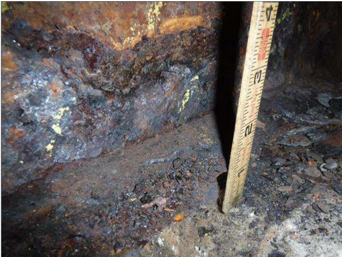
Span 4 Beam 10: 100 % SECTION LOSS BENT 3 BOTTOM FLANGE 1.5 IN WIDE X 3 FOOT LONG 5/16 IN REMAINING WEB 2 IN HIGH PRIORITY MAINTENANCE ISSUED
