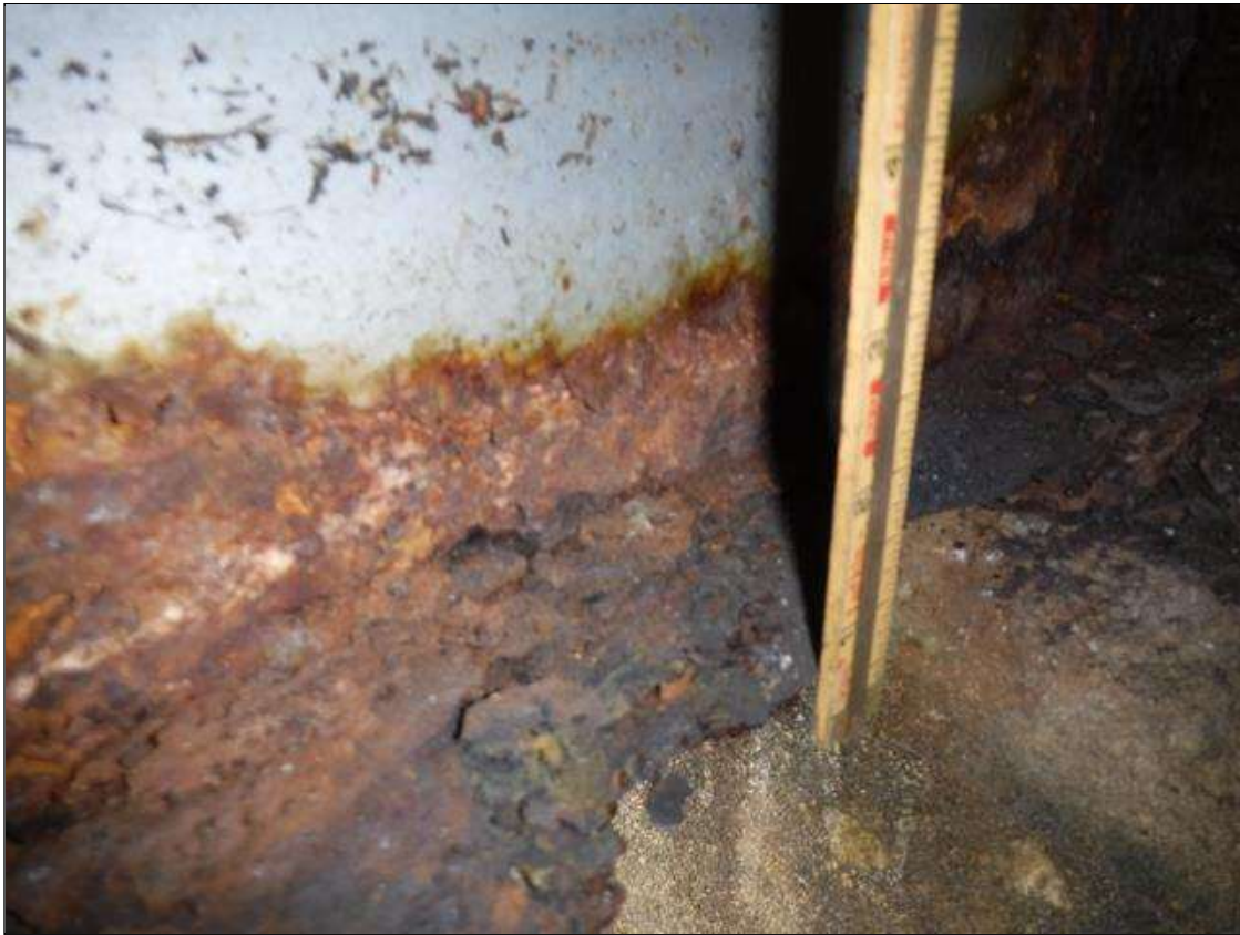
Span 3 Beam 1: SECTION LOSS 100 % BENT 3 BOTTOM FLANGE 1 IN WIDE X 2 FOOT LONG , WEB 5/16 IN REMAINING 4 IN HIGH PRIORITY MAINTENANCE ISSUED
