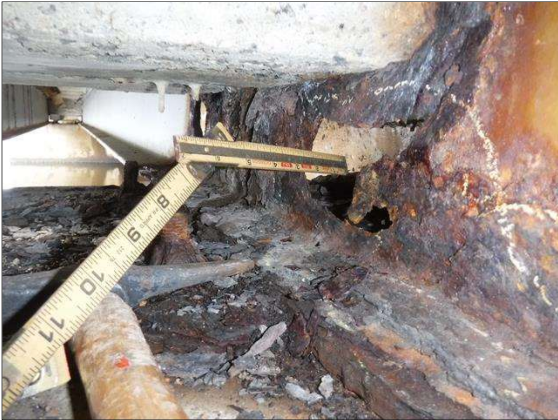
Span 3 Beam 9: SECTION LOSS BENT 2 WEB - HOLE 3 IN X 5 IN , SECTION LOSS BOTTOM FLANGE 100 % 1 IN WIDE X 3 FOOT LONG PRIORITY MAINTENANCE ISSUED
