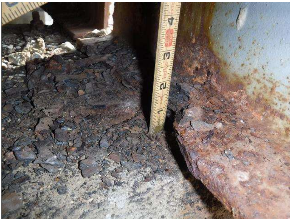
Span 1 Beam 10: SECTION LOSS BOTTOM FLANGE BENT 1 100 % 1 IN WIDE 16 IN LONG PRIORITY MAINTENANCE ISSUED
