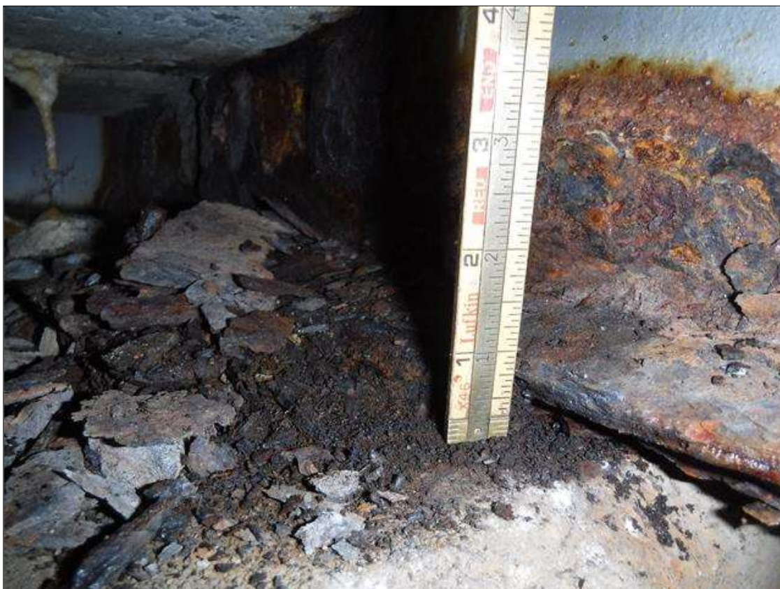
Span 4 Beam 2: 100 % SECTION LOSS EDGE BOTTOM FLANGE BENT 4 - 1 IN WIDE X 3 FOOT LONG PRIORITY MAINTENANCE ISSUED
