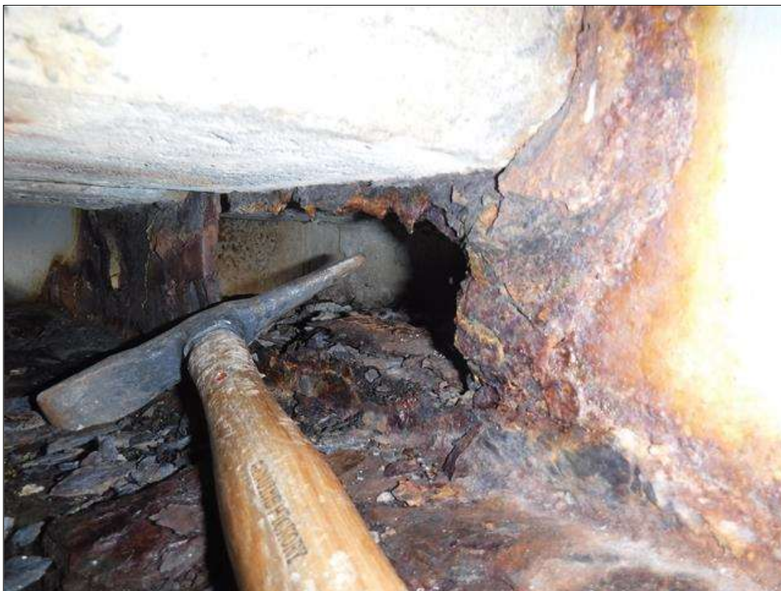
Span 1 Beam 2: SECTION LOSS WEB BENT 1 HOLE 4 IN HIGH X 8 IN LONG IN END, BOTTOM FLANGE 100 % SECTION LOSS 3/4 IN WIDE X 16 IN LONG PRIORITY MAINTENANCE ISSUED
