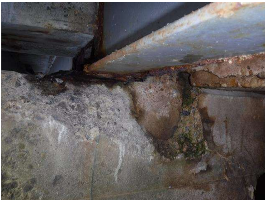
Bent 1 Cap 1: 10" X 20" LONG SPALL IN FACE OF CAP UNDER BEAM 2 SPAN 1 SIDE
