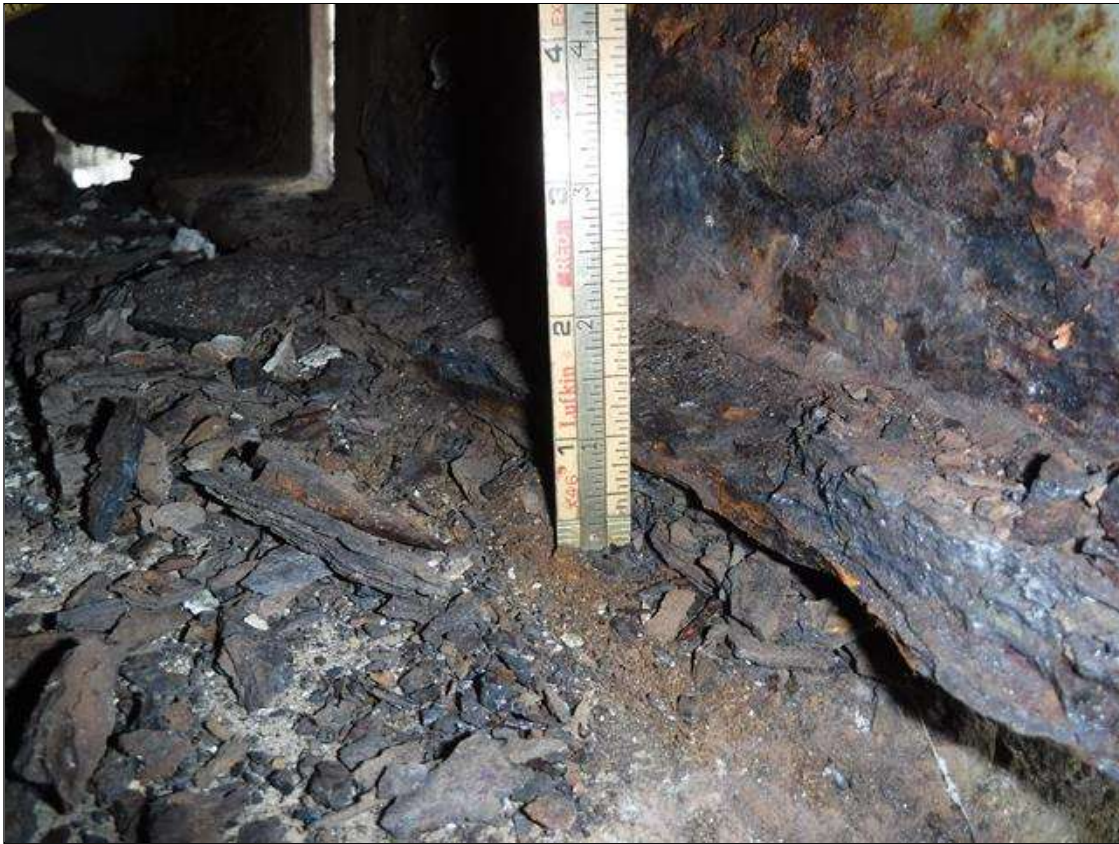
Span 3 Beam 1: SECTION LOSS EDGE BENT 2 BOTTOM FLANGE 100 % -1 IN WIDE X 2 FOOT LONG , 5/16 IN REMAINING WEB 2 IN HIGH PRIORITY MAINTENANCE ISSUED
