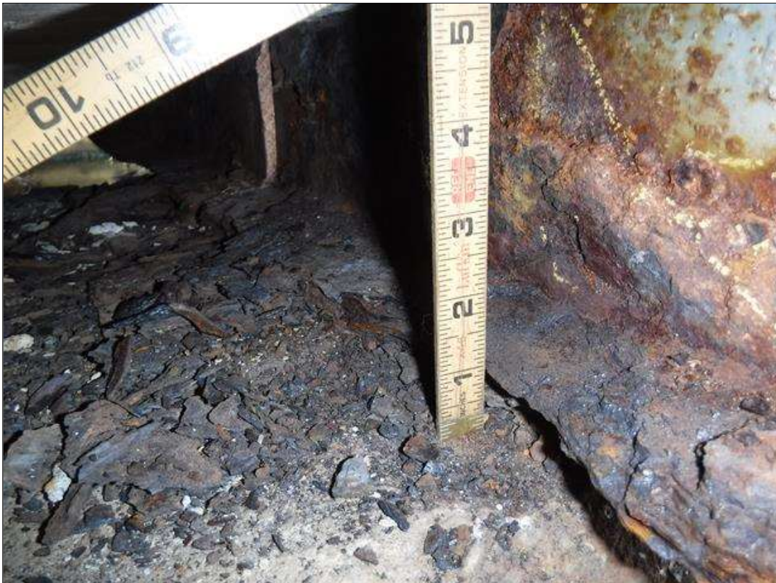
Span 2 Beam 1: SECTION LOSS EDGE BOTTOM FLANGE BENT 1 KNIFE EDGE 1/16 IN REMAINING, 5/16 IN REMAINING WEB 5 IN HIGH PRIORITY MAINTENANCE ISSUED
