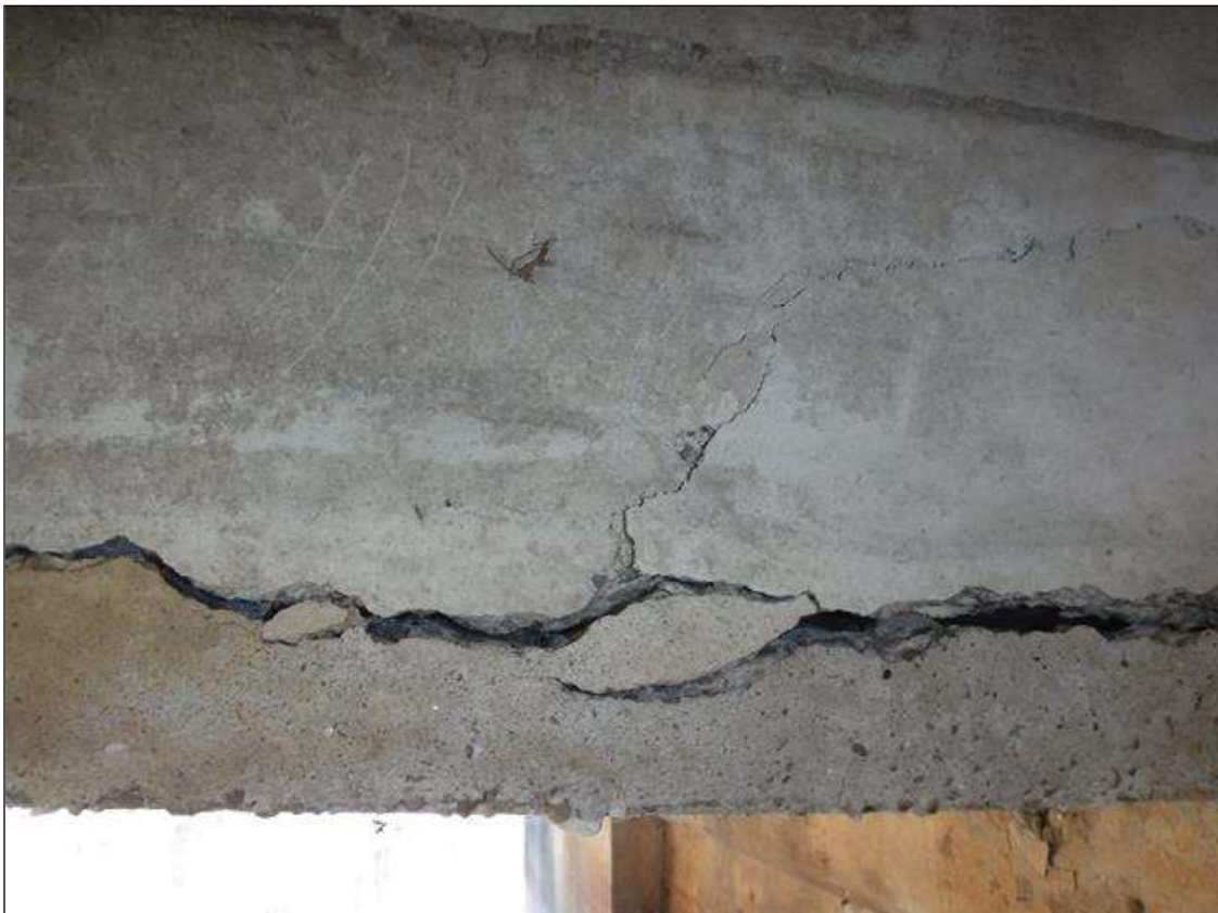
CRACKING IN CONCRETE INCASEMENT BEAM 6 SPAN 5 AT BENT 4
