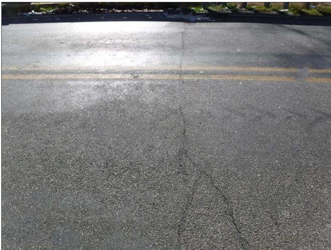
Span 1 Wearing Surface: TRANSVERSE CRACK END BENT 1
