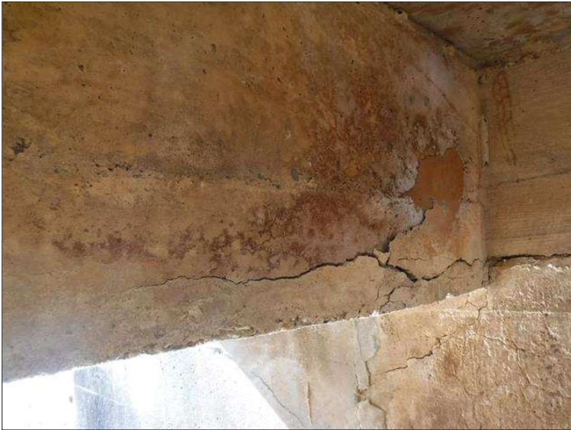
4' OF CRACKING IN CONCRETE INCASEMENT
