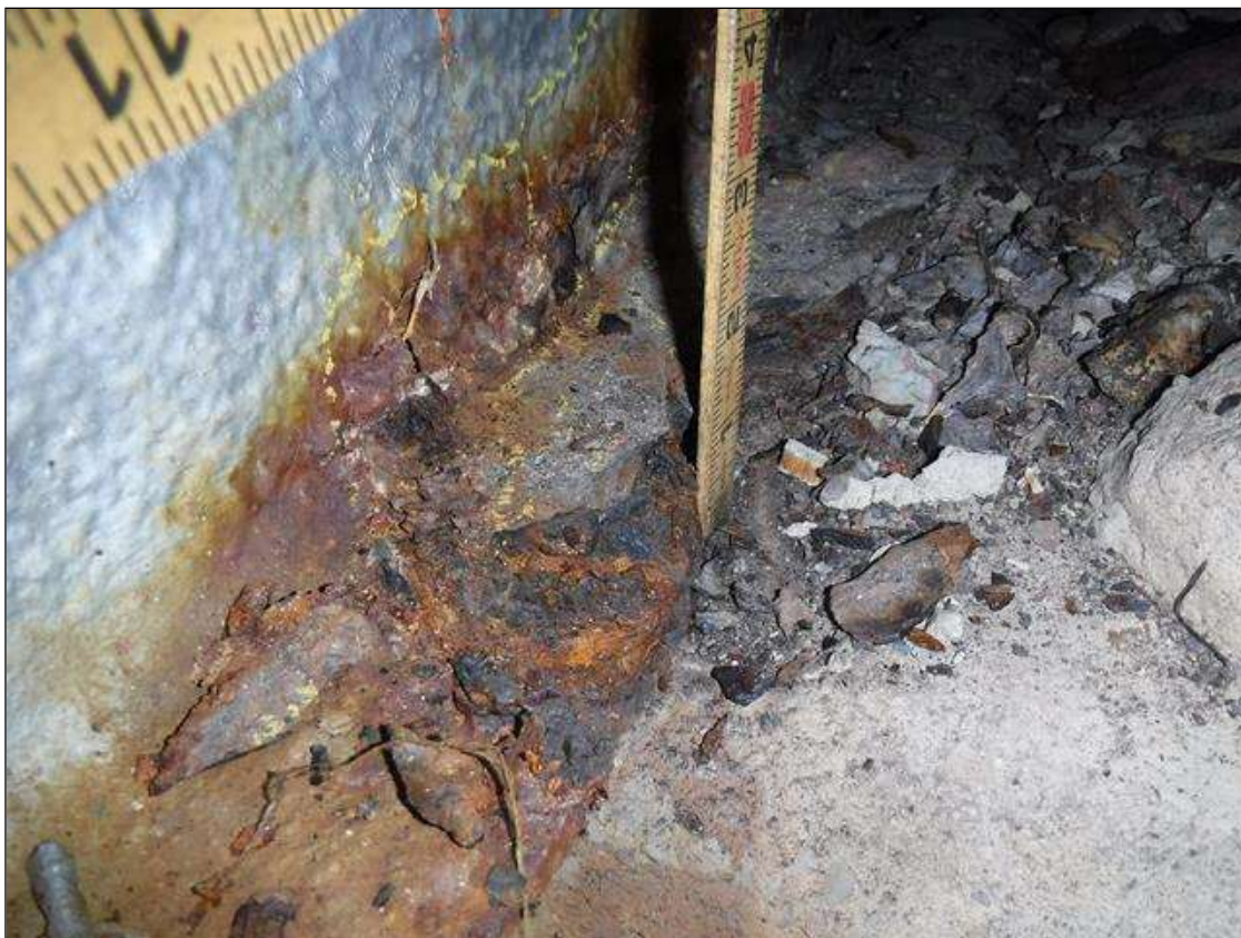
Span 5 Beam 9: SECTION LOSS WEB BENT 4 -1 IN DIAMETER OVER BEARING , SECTION LOSS BOTTOM FLANGE 100 % IN EDGE 1 IN WIDE X 6 IN LONG BEARING OUT, PRIORITY MAINTENANCE ISSUED
