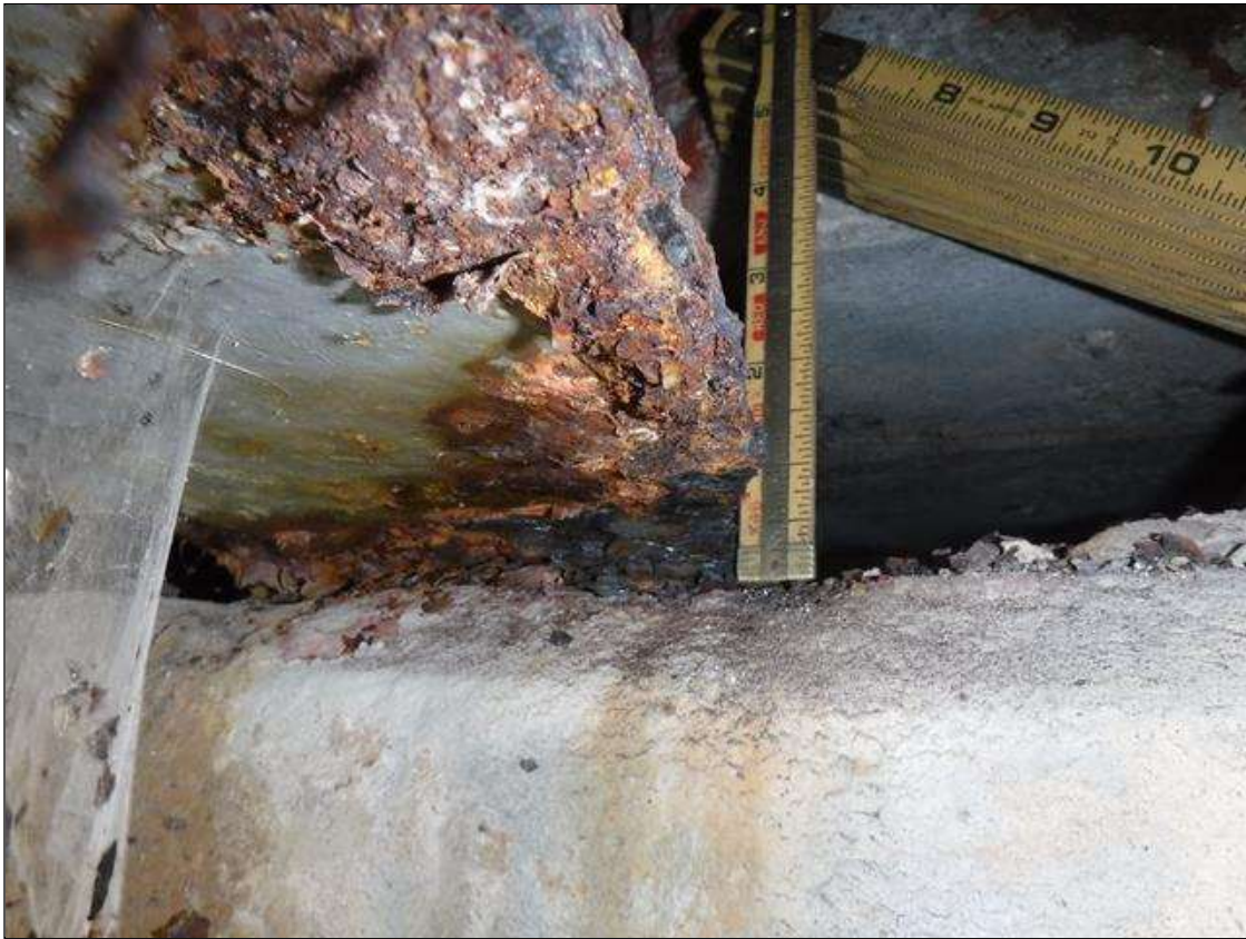
Span 3 Beam 2: SECTION LOSS BOTTOM FLANGE BENT 3 - 1/4 IN REMAINING IN EDGE 14 IN LONG , 5/16 IN REMAINING WEB 5 IN HIGH PRIORITY MAINTENANCE ISSUED
