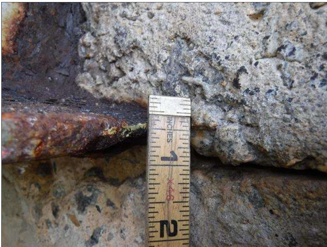
Span 1 Beam 1: SECTION LOSS BOTTOM FLANGE 1/4 IN REMAINING 2 IN LONG AT ABUTMENT 1 PRIORITY MAINTENANCE ISSUED
