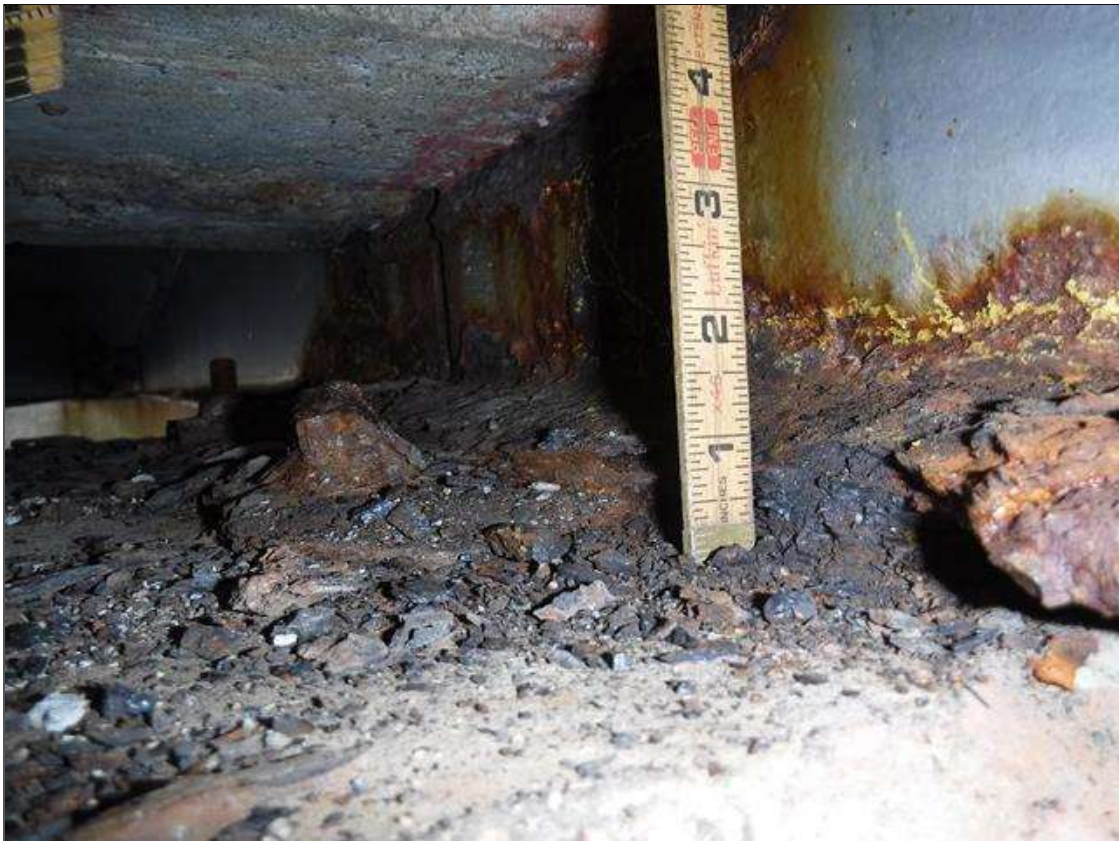
Span 2 Beam 2: SECTION LOSS BOTTOM FLANGE BENT 2 - 100 % 1.5 IN WIDE X 14 IN LONG , 1/4 IN REMAINING WEB 2 IN HIGH PRIORITY MAINTENANCE ISSUED
