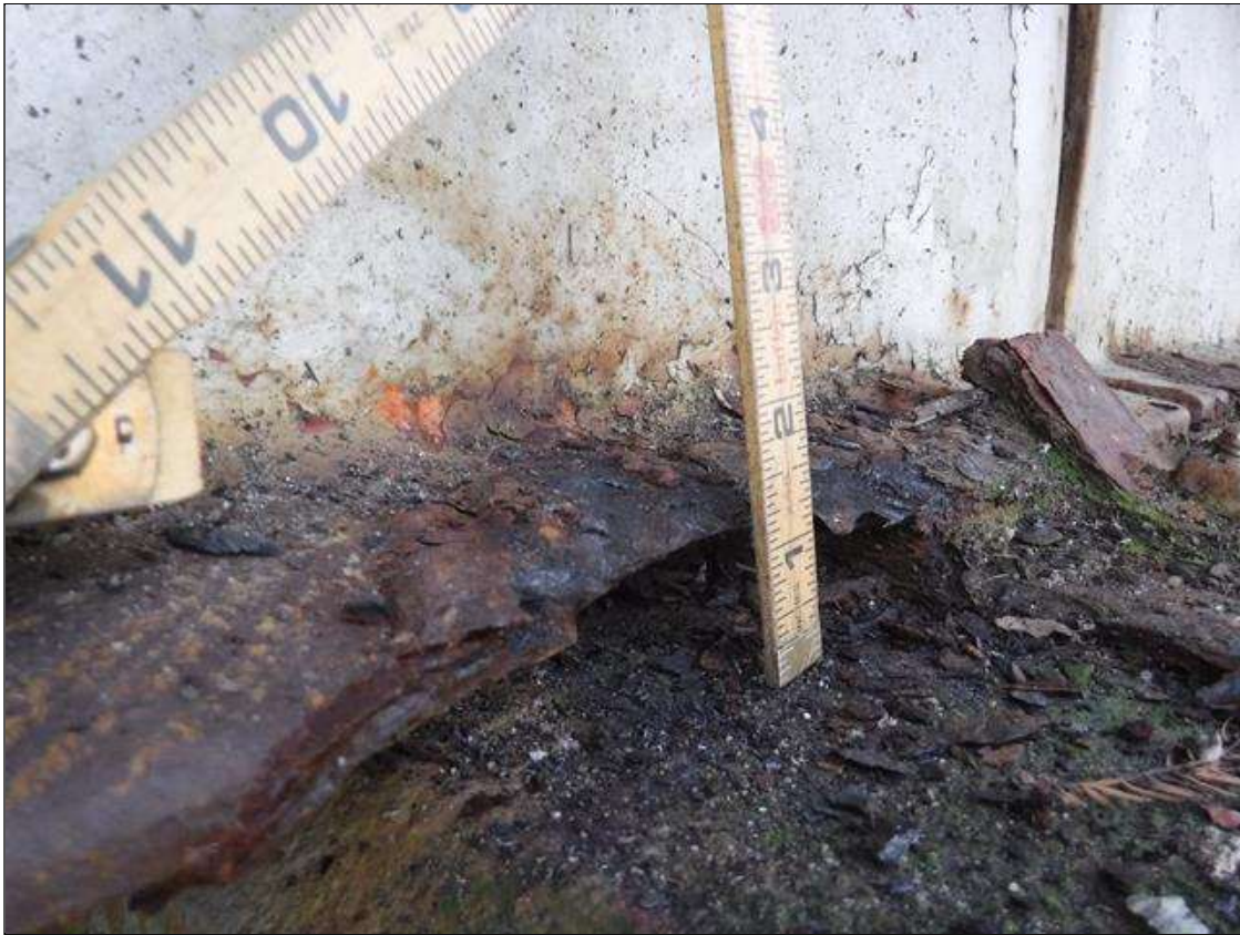
Span 5 Beam 1: SECTION LOSS AT BENT 4 BOTTOM FLANGE 100 % 1 IN WIDE X 6 IN LONG , WEB 3/16 IN REMAINING 3 IN HIGH X 1 FOOT LONG PRIORITY MAINTENANCE ISSUED
