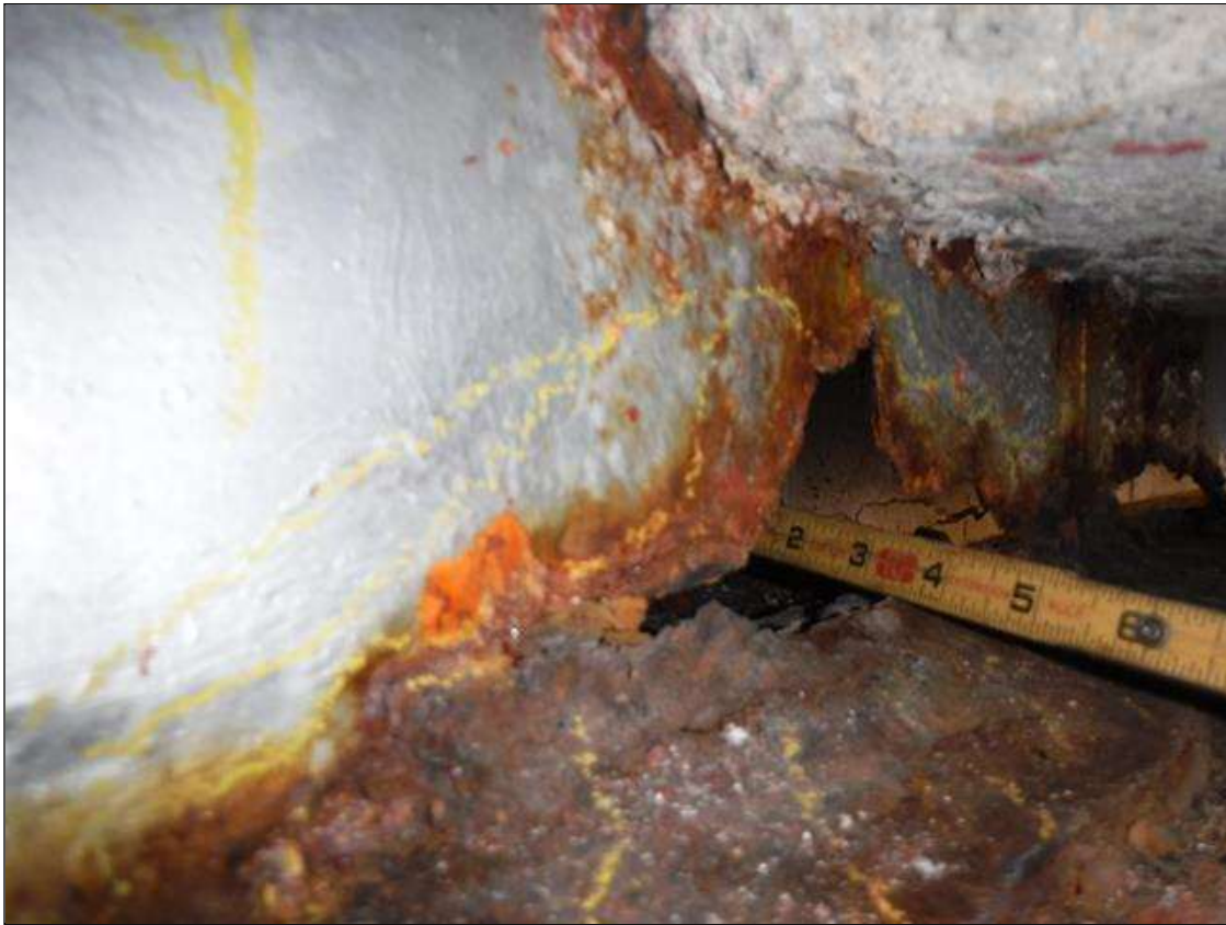
Span 5 Beam 2: SECTION LOSS WEB BENT 4 - 3 IN HIGH X 8 IN LONG HOLE 1 IN UP FROM BOTTOM FLANGE OVER BEARING, SECTION LOSS 100 % BOTTOM FLANGE 1 IN WIDE X 8 IN LONG FROM BEARING OUT PRIORITY MAINTENANCE ISSUED
