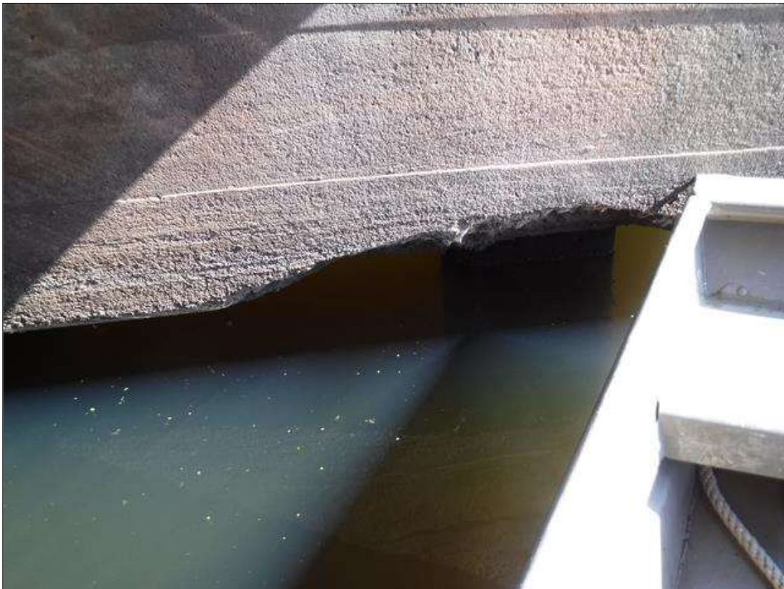
4' LONG X 6" WIDE SPALL IN BOTTOM CORNER OF BENT 2 CAP WITH EXPOSED STEEL
