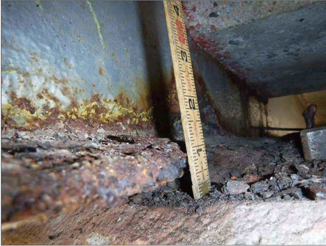
Span 2 Beam 9: 100 % SECTION LOSS BOTTOM FLANGE BENT 1 EDGE 3/4 IN WIDE X 12 IN LONG , 1/4 REMAINING MIDDLE BOTTOM FLANGE , 5/16 IN REMAINING WEB 3 IN HIGH PRIORITY MAINTENANCE ISSUED
