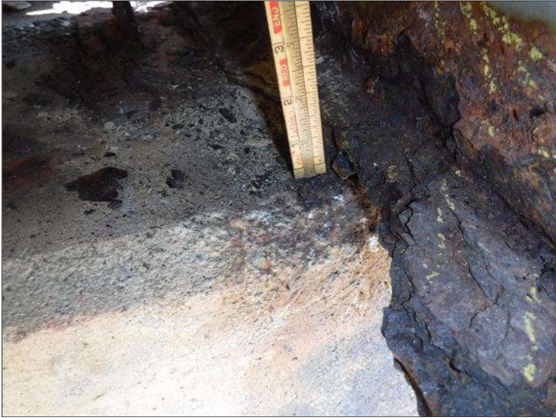
Span 4 Beam 10: SECTION LOSS AT BENT 4 EDGE BOTTOM FLANGE 100 % 18 IN LONG X 2 IN WIDE , WEB 4 IN HIGH 5/16 IN REMAINING PRIORITY MAINTENANCE ISSUED
