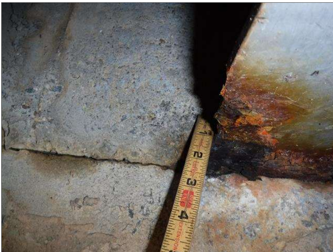
Span 1 Beam 2: BOTTOM FLANGE AT ABUTMENT 1 100 % SECTION LOSS 3/4 IN WIDE X 2 IN LONG PRIORITY MAINTENANCE ISSUED
