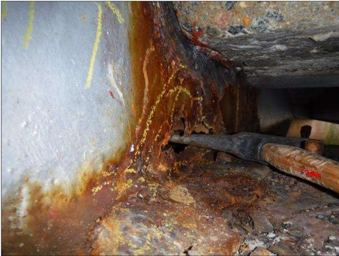
Span 2 Beam 2: SECTION LOSS AT BENT 1 WEB 100 % HOLE 1 IN HIGH X 4 IN LONG 1 IN UP FROM BOTTOM FLANGE AND 100 % IN BOTTOM FLANGE 1.5 IN WIDE X 12 IN LONG PRIORITY MAINTENANCE ISSUED
