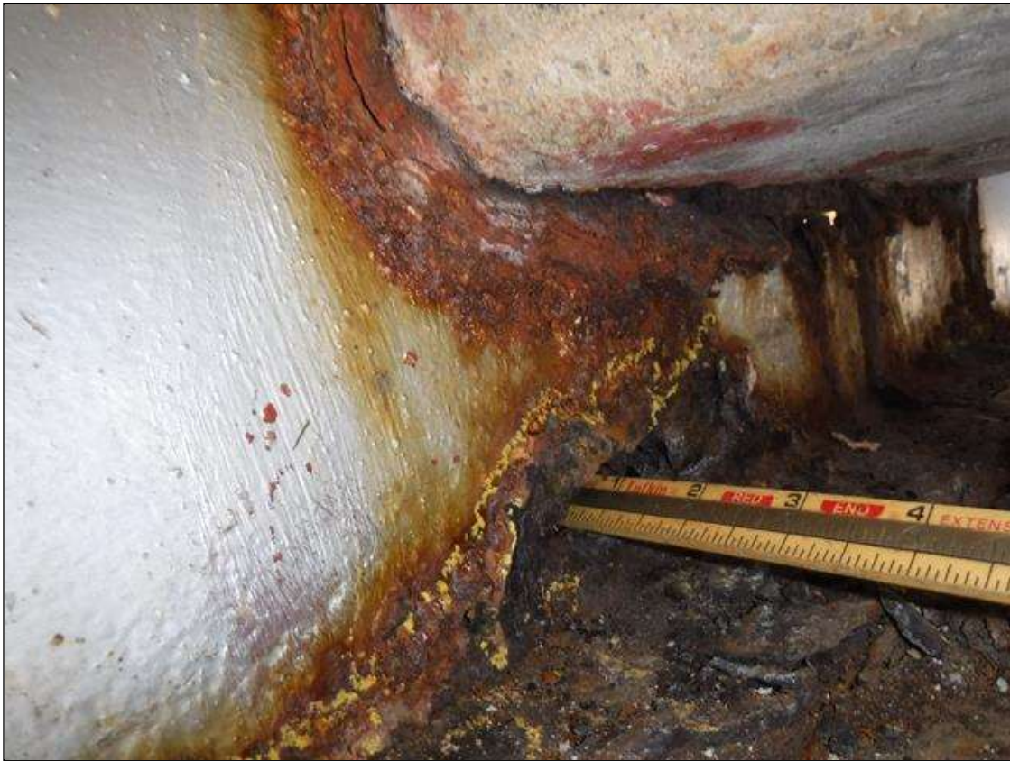
Span 2 Beam 9: SECTION LOSS BENT 2 WEB - HOLE 1 IN DIAMETER 1 IN UP FROM BOTTOM FLANGE, 100 % SECTION LOSS IN EDGE BOTTOM FLANGE 1 IN WIDE X 12 IN LONG, 1/4 IN REMAINING IN MIDDLE BOTTOM FLANGE PRIORITY MAINTENANCE ISSUED
