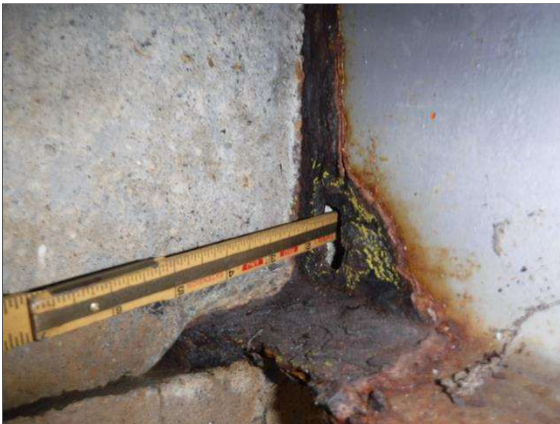
Span 5 Beam 2: SECTION LOSS WEB ABUTMENT 2 WITH HOLE 1.5 IN DIAMETER 1 IN UP FROM BOTTOM FLANGE 1/2 IN FROM ABUTMENT WALL, SECTION LOSS BOTTOM FLANGE 100 % 3/4 IN WIDE X 3 IN LONG PRIORITY MAINTENANCE ISSUED
