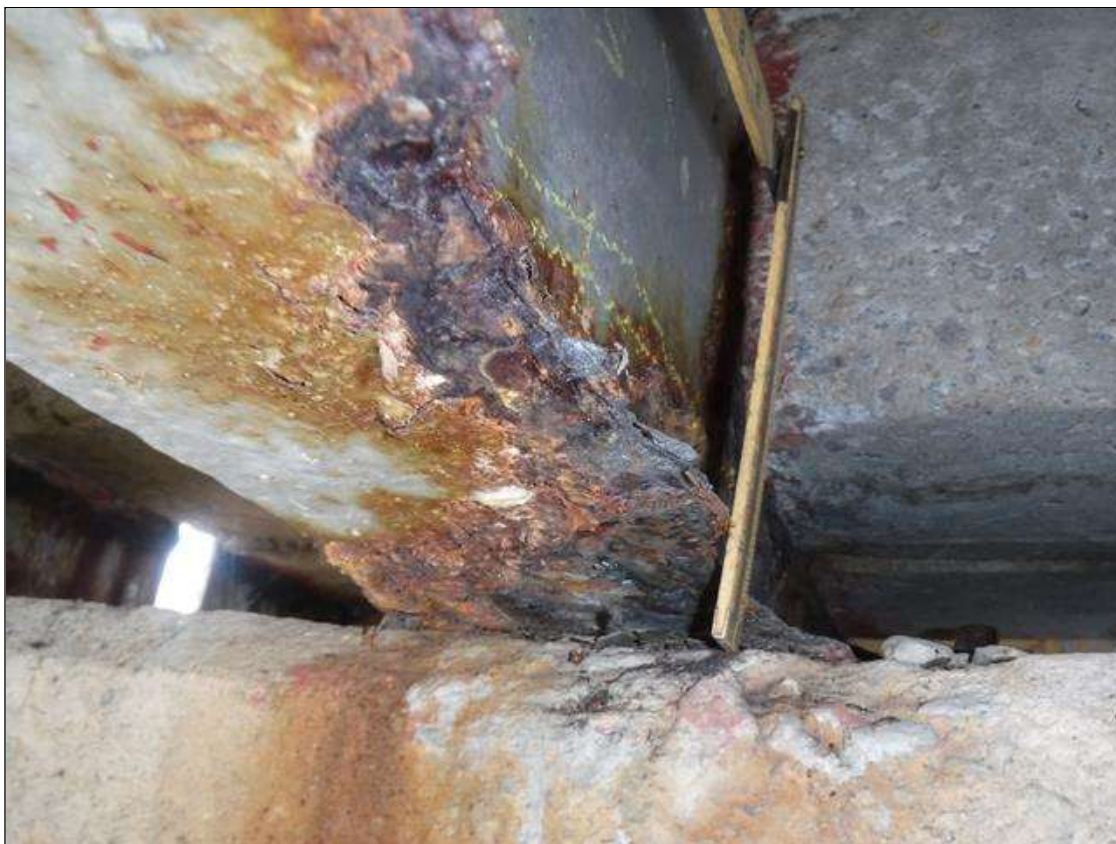
Span 4 Beam 9: SECTION LOSS EDGE BOTTOM FLANGE AT BENT 3 -100 % 1 IN WIDE X 15 IN LONG, WEB 5/16 IN REMAINING 2 IN HIGH PRIORITY MAINTENANCE ISSUED
