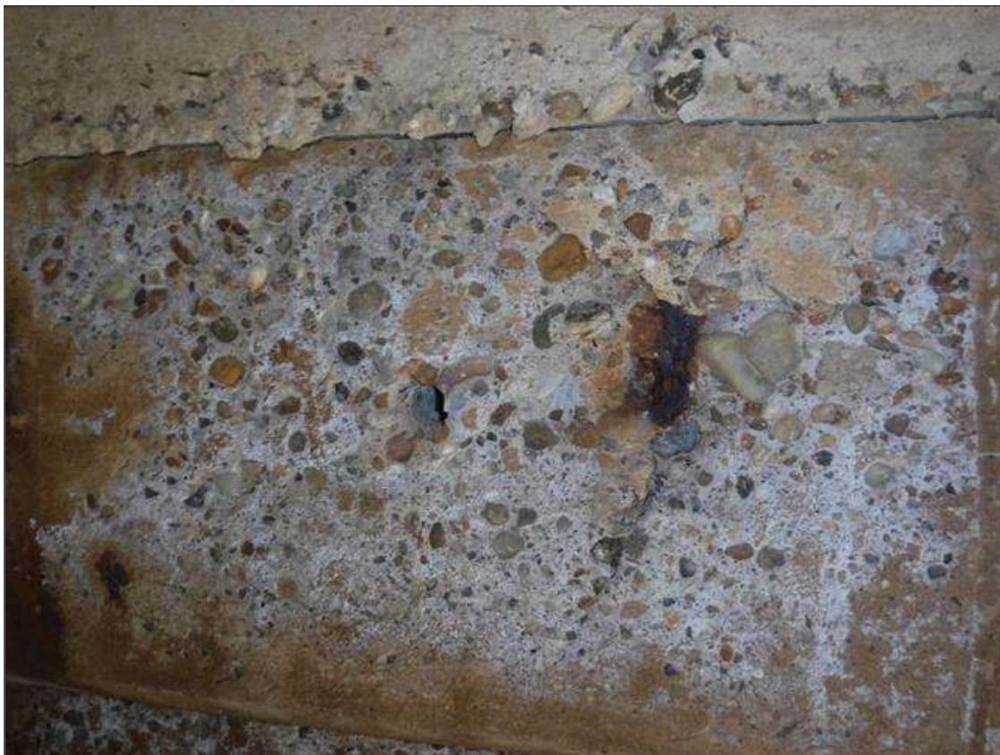
SURFACE SPALL IN BENT 1 CAP SPAN 1 SIDE WITH EXPOSED STEEL
