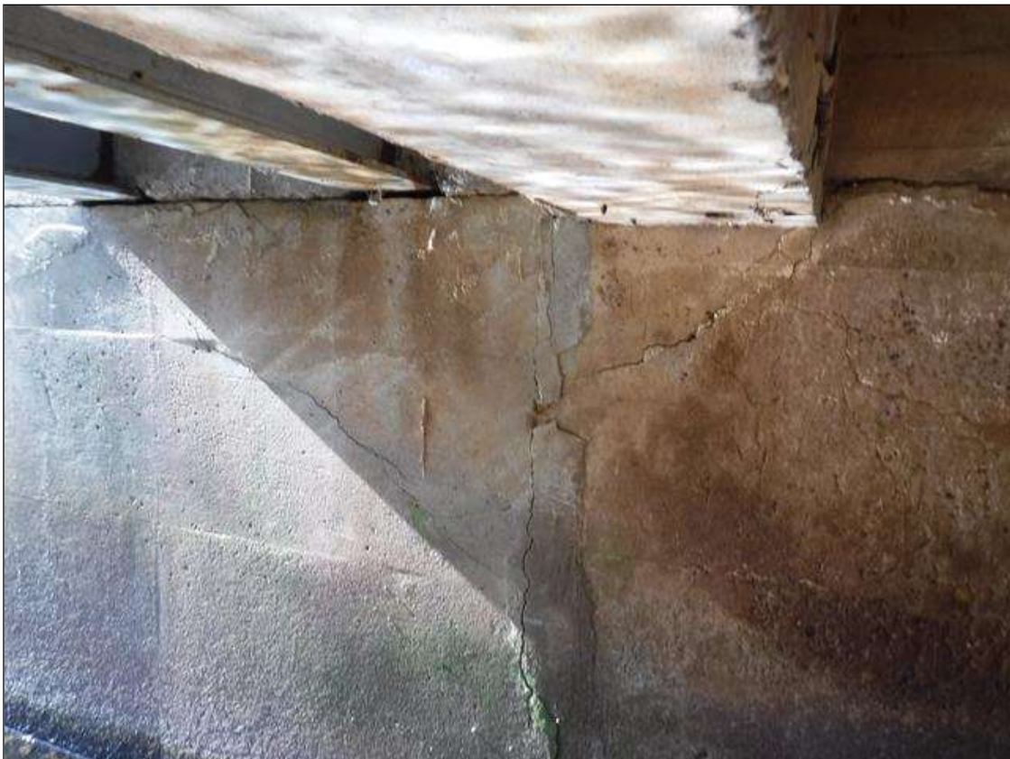
End Bent 1 Abutment/Backwall : MAP CRACKING IN FACE
