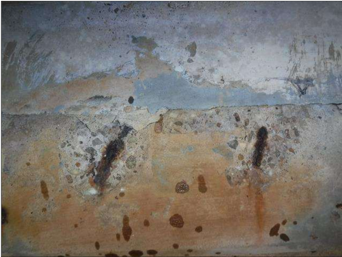
SPALL WITH EXPOSED STEEL IN BENT 4 CAP SPAN 5 SIDE
