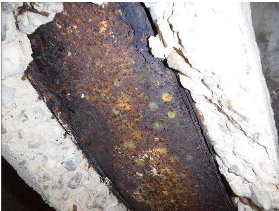
Span 5 Beam 7: RUST ON BOTTOM FLANGE
