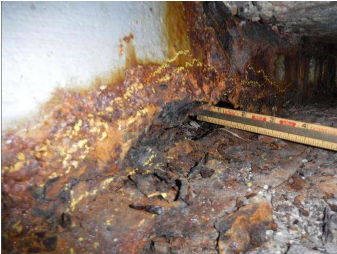
Span 3 Beam 2: SECTION LOSS WEB BENT 2 HOLE 4 IN DIAMETER 1 IN UP FROM BOTTOM FLANGE 1 FOOT FROM END , 100 % SECTION LOSS BOTTOM FLANGE 1 IN WIDE X 1 FOOT LONG PRIORITY MAINTENANCE ISSUED
