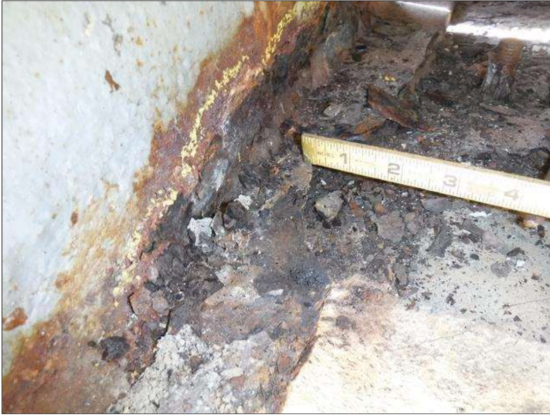
Span 2 Beam 10: SECTION LOSS BOTTOM FLANGE BENT 1 -100 % 1.5 IN WIDE X 12 IN LONG , 1/4 IN REMAINING WEB 5 IN HIGH PRIORITY MAINTENANCE ISSUED
