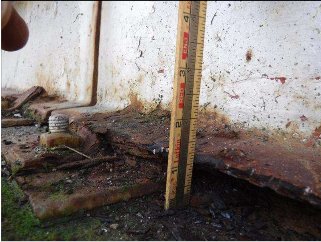
Span 4 Beam 1: SECTION LOSS BOTTOM FLANGE AT BENT 4 -100 % IN EDGE 1 IN WIDE X 2 FOOT LONG , WEB 5/16 IN REMAINING 3 IN HIGH PRIORITY MAINTENANCE ISSUED
