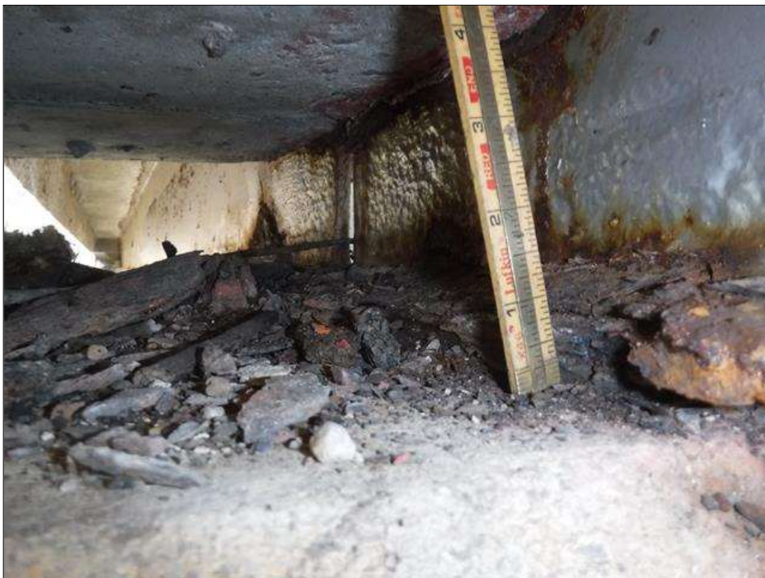
Span 1 Beam 9: SECTION LOSS 100 % BOTTOM FLANGE AT BENT 1 - 3/4 IN X 12 IN LONG , SECTION LOSS WEB 3 IN HIGH X 5/16 IN REMAINING PRIORITY MAINTENANCE ISSUED
