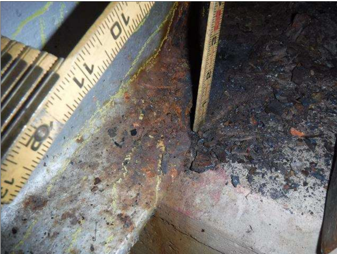
Span 4 Beam 2: SECTION LOSS BOTTOM FLANGE BENT 3 - 100 % IN EDGE 1 IN WIDE X 12 IN LONG 5/16 IN REMAINING MIDDLE, SECTION LOSS WEB 5/16 IN REMAINING 4 IN HIGH PRIORITY MAINTENANCE ISSUED
