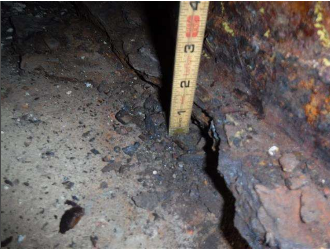
Span 4 Beam 1: SECTION LOSS BOTTOM FLANGE AT BENT 3 -100 % EDGE 1.5 IN WIDE X 2 FOOT LONG , WEB 5/16 IN REMAINING 4 IN HIGH PRIORITY MAINTENANCE ISSUED
