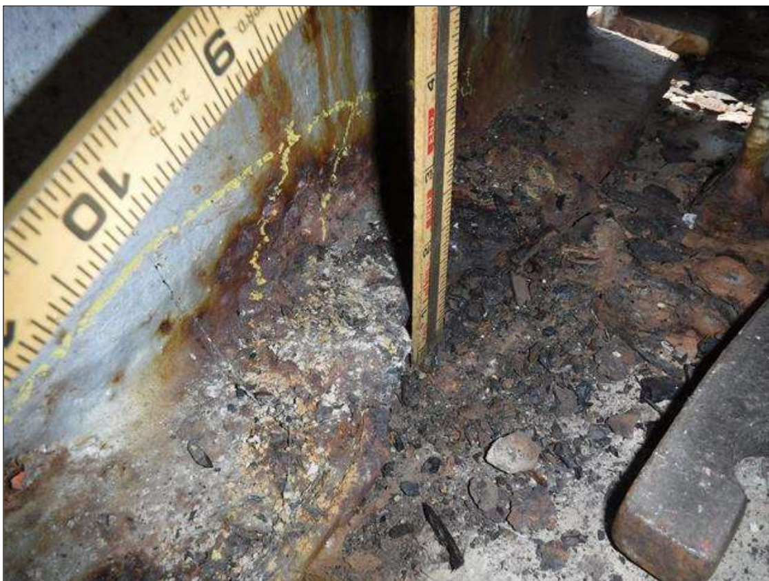
Span 4 Beam 10: SECTION LOSS IN EDGE BOTTOM FLANGE AT BENT 3 - 100 % 1/2 IN WIDE X 11 IN LONG PRIORITY MAINTENANCE ISSUED
