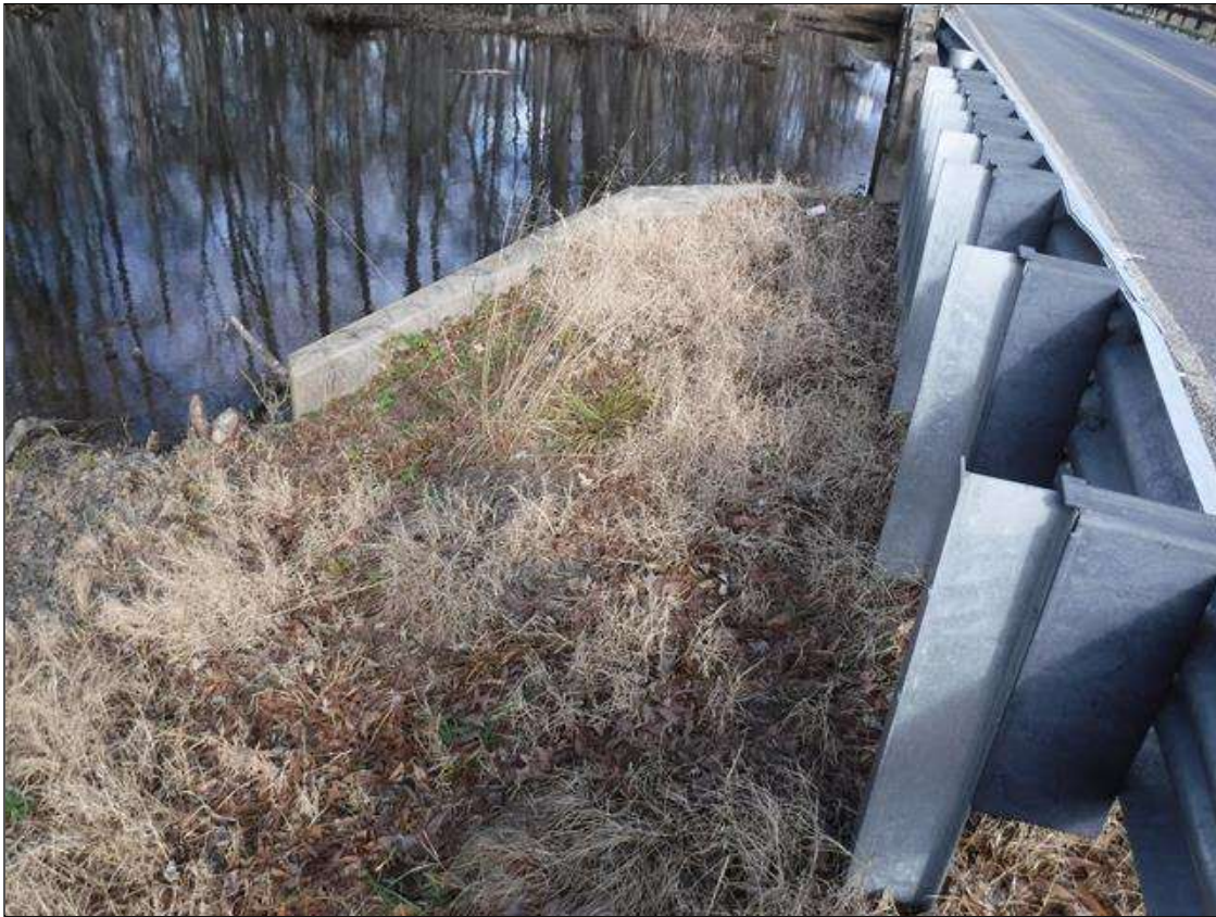
MISSING DELINEATOR SOUTH WEST CORNER SIMILAR AT NORTH EAST CORNER PRIORITY MAINTENANCE ISSUED
