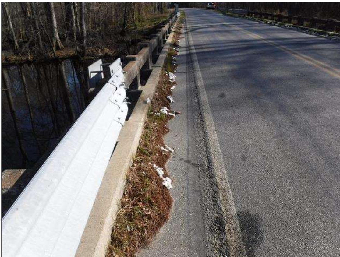
DEBRIS ALONG GUARDRAIL
