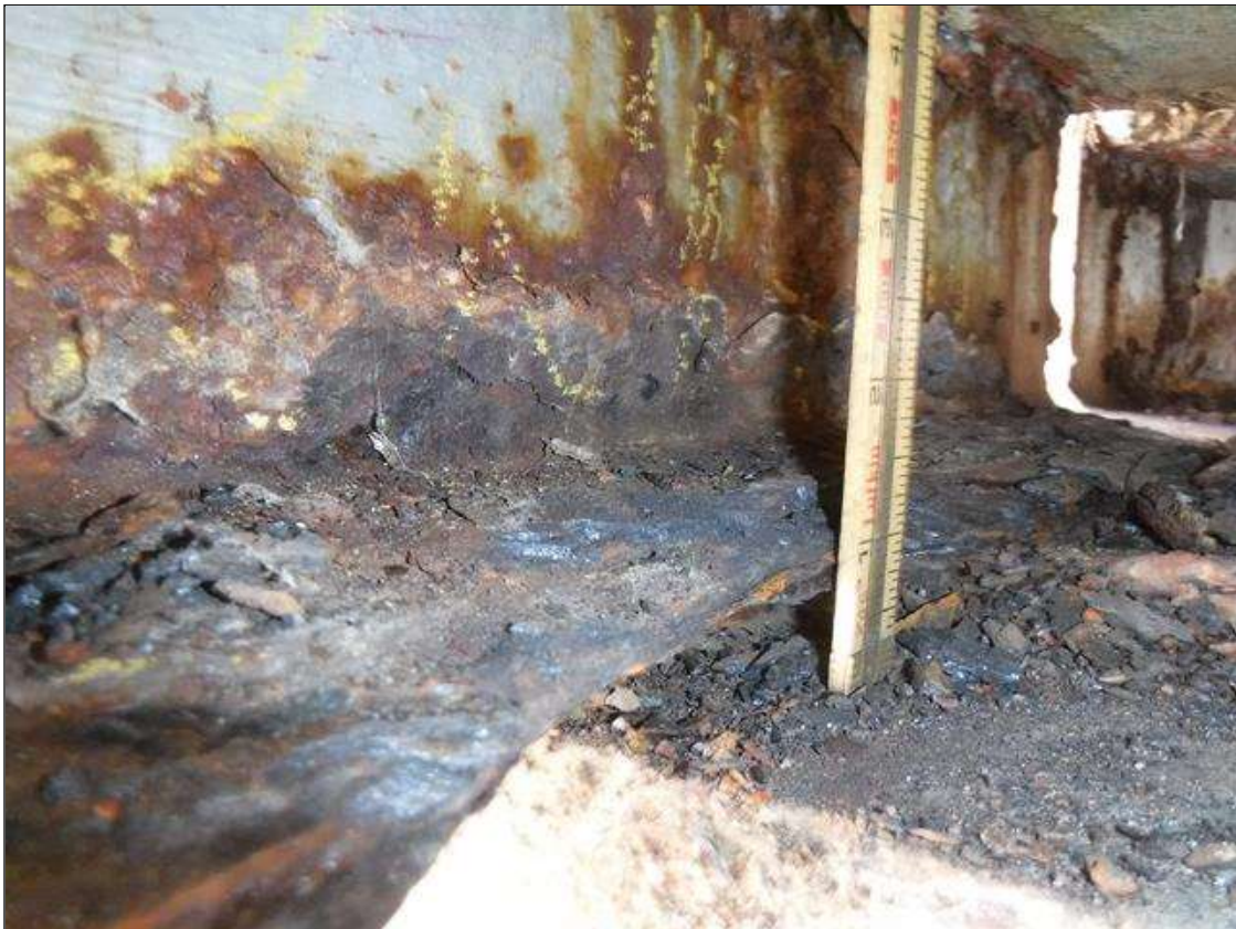
Span 3 Beam 1: SECTION LOSS BOTTOM FLANGE BENT 3 - 100 % EDGE 1 IN WIDE X 1 FOOT LONG , 3/8 IN REMAINING WEB PRIORITY MAINTENANCE ISSUED
