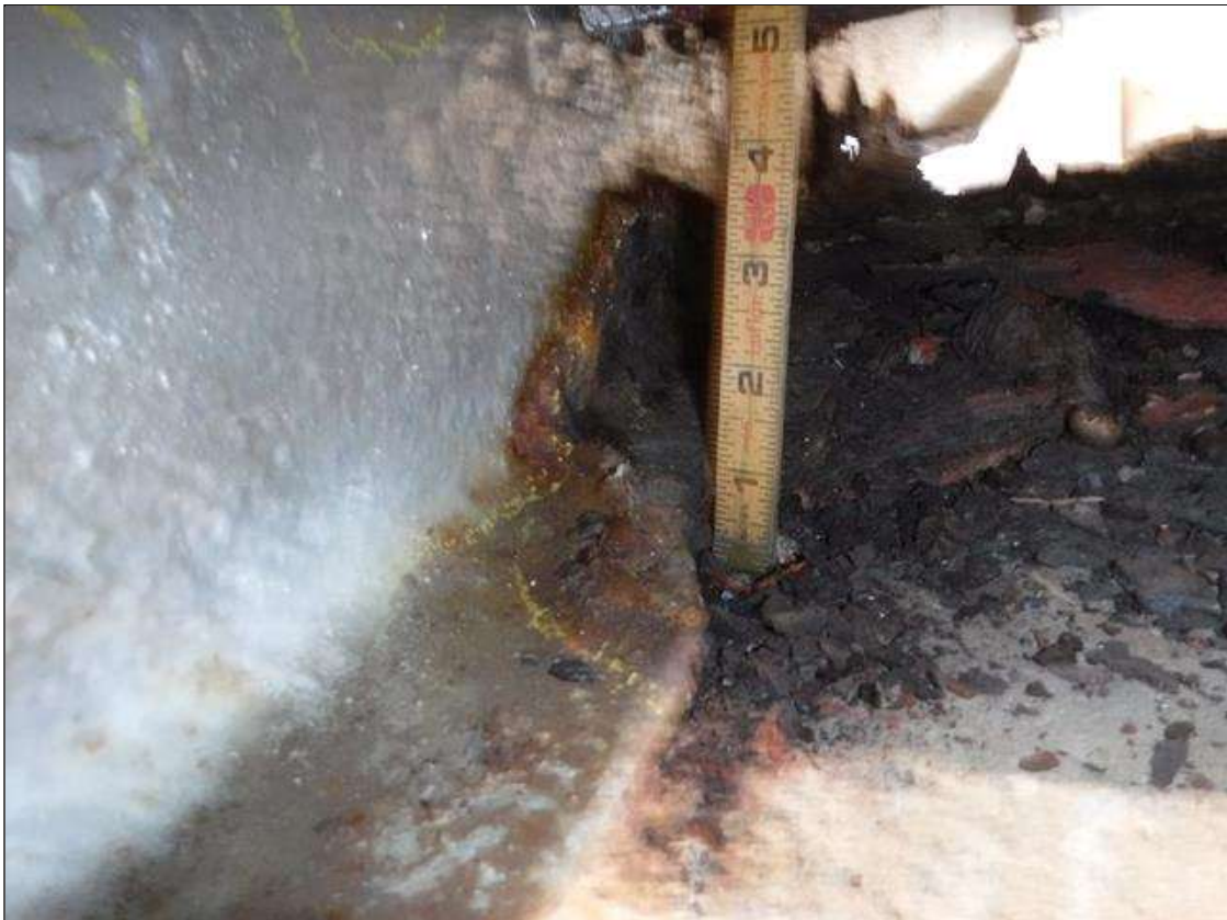
Span 1 Beam 2: SECTION LOSS BOTTOM FLANGE BENT 1 100 % 1 IN WIDE X 16 IN LONG , SECTION LOSS WEB 5/16 IN REMAINING 2 IN HIGH X 6 IN LONG PRIORITY MAINTENANCE ISSUED
