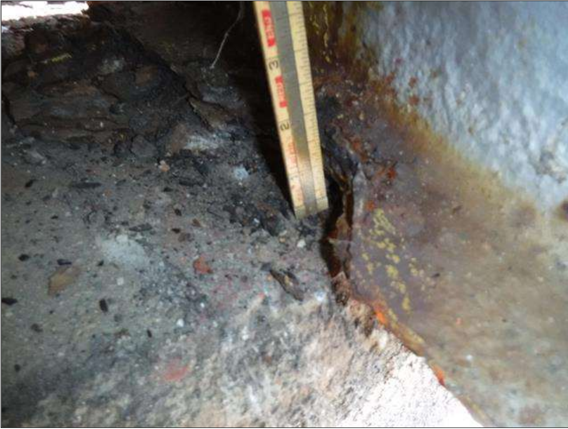
Span 3 Beam 10: SECTION LOSS BOTTOM FLANGE BENT 3 - 100 % IN EDGE 2 IN WIDE X 1 FOOT LONG , WEB 5/16 IN REMAINING 2 IN HIGH PRIORITY MAINTENANCE ISSUED
