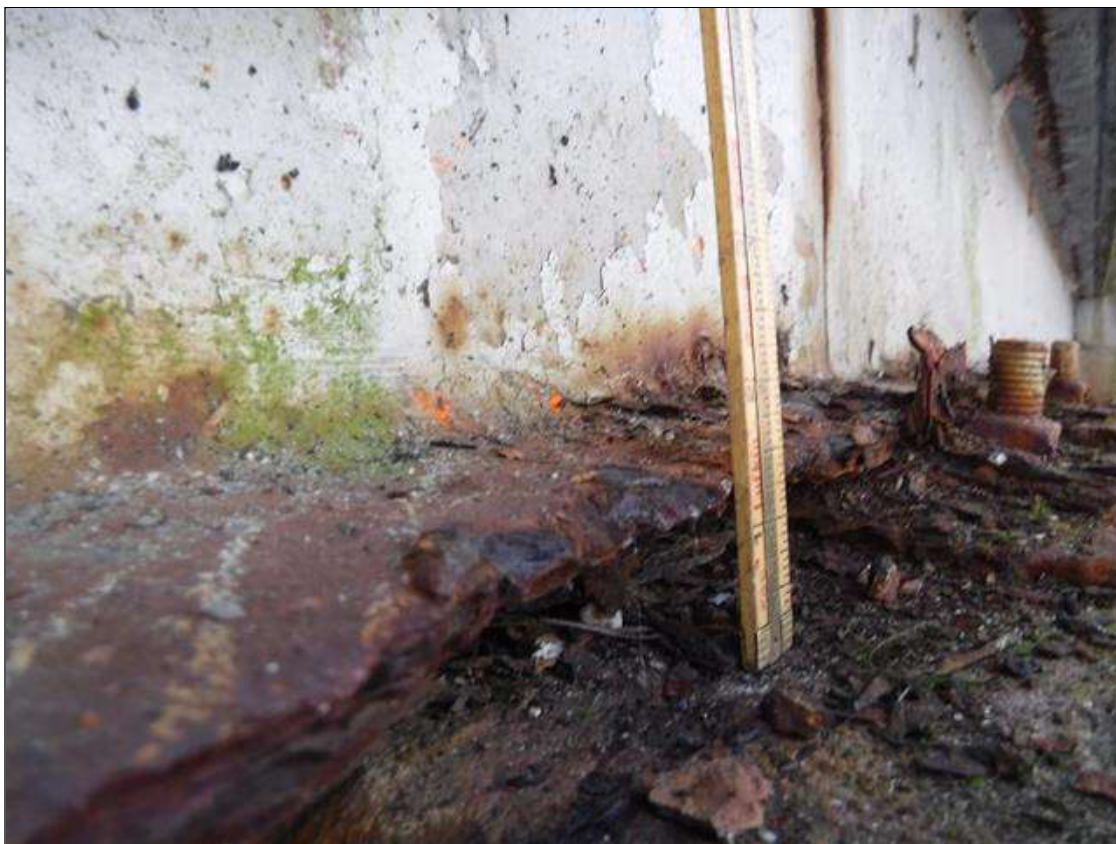
Span 2 Beam 1: 100 % SECTION LOSS BOTTOM FLANGE AT BENT 1 - 1.5 IN WIDE X 14 IN LONG , 5/16 IN REMAINING IN WEB 5 IN HIGH X 1 FOOT LONG PRIORITY MAINTENANCE ISSUED
