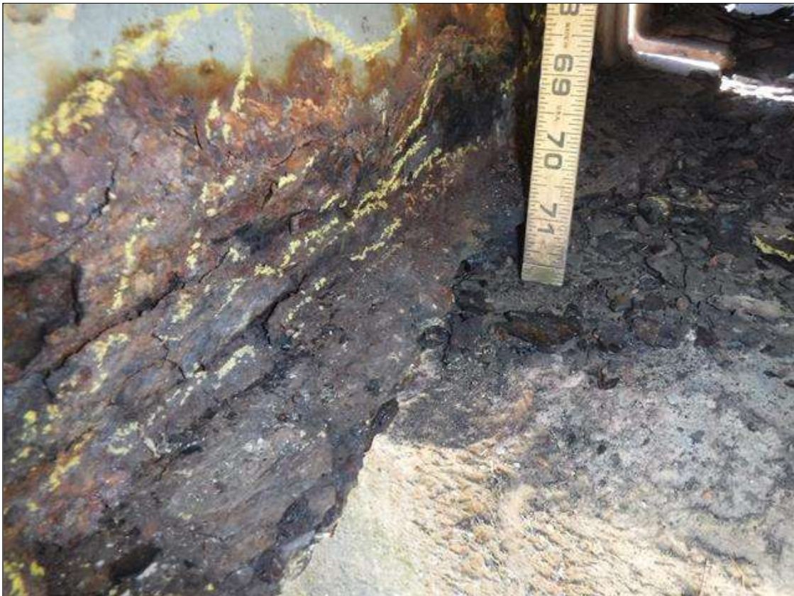
Span 3 Beam 10: SECTION LOSS BOTTOM FLANGE BENT 2 - 100 % IN EDGE 1.5 IN WIDE X 2 FOOT LONG , 5/16 IN REMAINING WEB 3 IN HIGH X 2 FOOT LONG PRIORITY MAINTENANCE ISSUED
