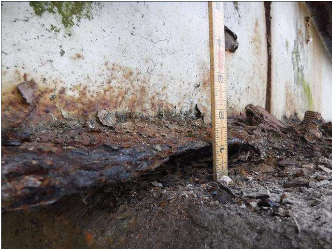
Span 3 Beam 1: SECTION LOSS BOTTOM FLANGE BENT 2 -100 % EDGE 1.5 IN WIDE X 2 FOOT LONG 1/4 IN RM IN MIDDLE BOTTOM FLANGE , 1/4 IN REMAINING WEB 4 IN HIGH X 4 FOOT PRIORITY MAINTENANCE ISSUED
