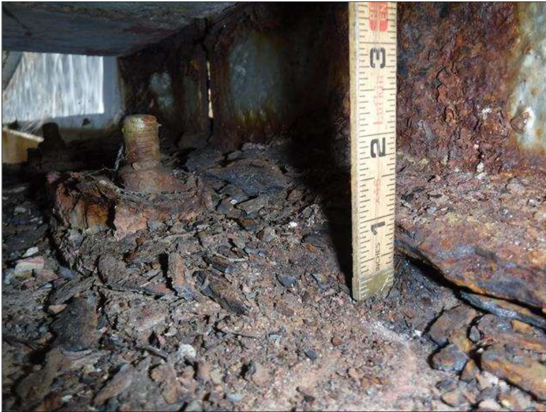
Span 3 Beam 9: SECTION LOSS BOTTOM FLANGE BENT 2 - 1/4 IN REMAINING 1 FOOT LONG , WEB 3/8 IN REMAINING 2 IN HIGH PRIORITY MAINTENANCE ISSUED
