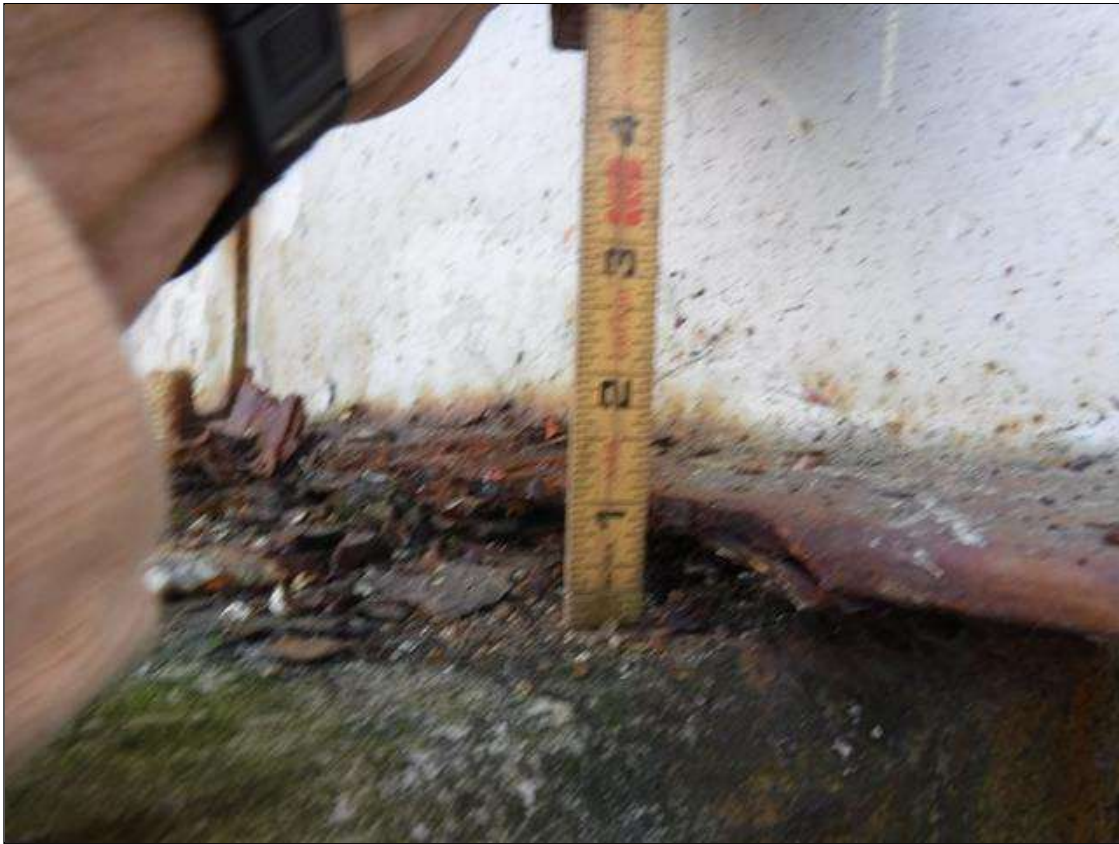
Span 1 Beam 1: 100 % SECTION LOSS BOTTOM FLANGE AT BENT 1 1 IN WIDE X 1.5 FOOT LONG AND 5/16 IN REMAINING IN WEB 5 IN HIGH X 1 FOOT LONG PRIORITY MAINTENANCE ISSUED
