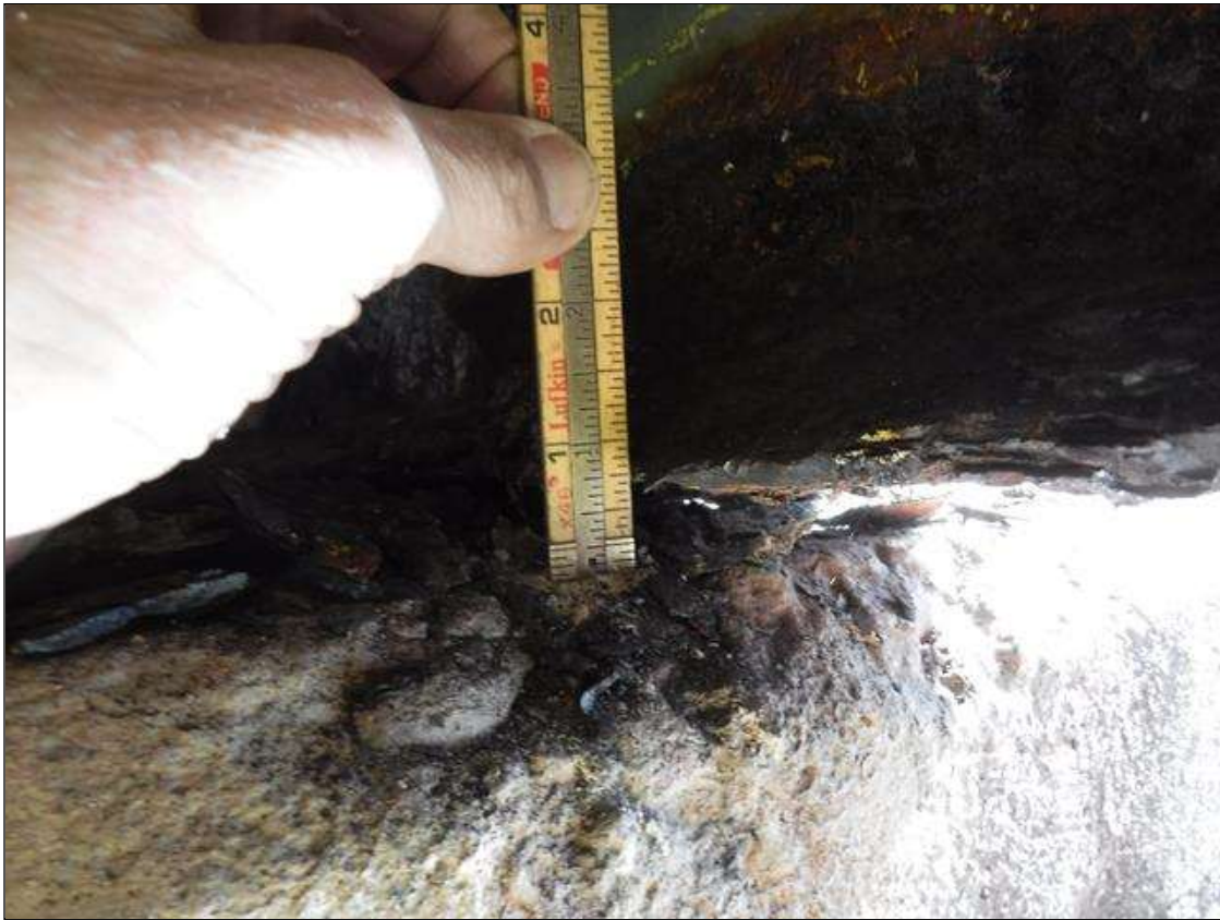
Span 2 Beam 10: SECTION LOSS BOTTOM FLANGE BENT 2 - 100 % EDGE 1.5 IN X 12 IN , 1/4 IN REMAINING WEB 3 IN HIGH PRIORITY MAINTENANCE ISSUED
