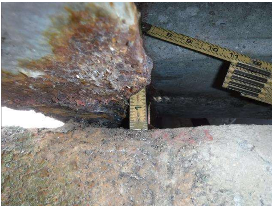
Span 2 Beam 1: 100 % SECTION LOSS BOTTOM FLANGE BENT 2- 1.5 IN WIDE X 10 IN LONG , SECTION LOSS WEB 3 IN HIGH X 1/4 IN REMAINING PRIORITY MAINTENANCE ISSUED
