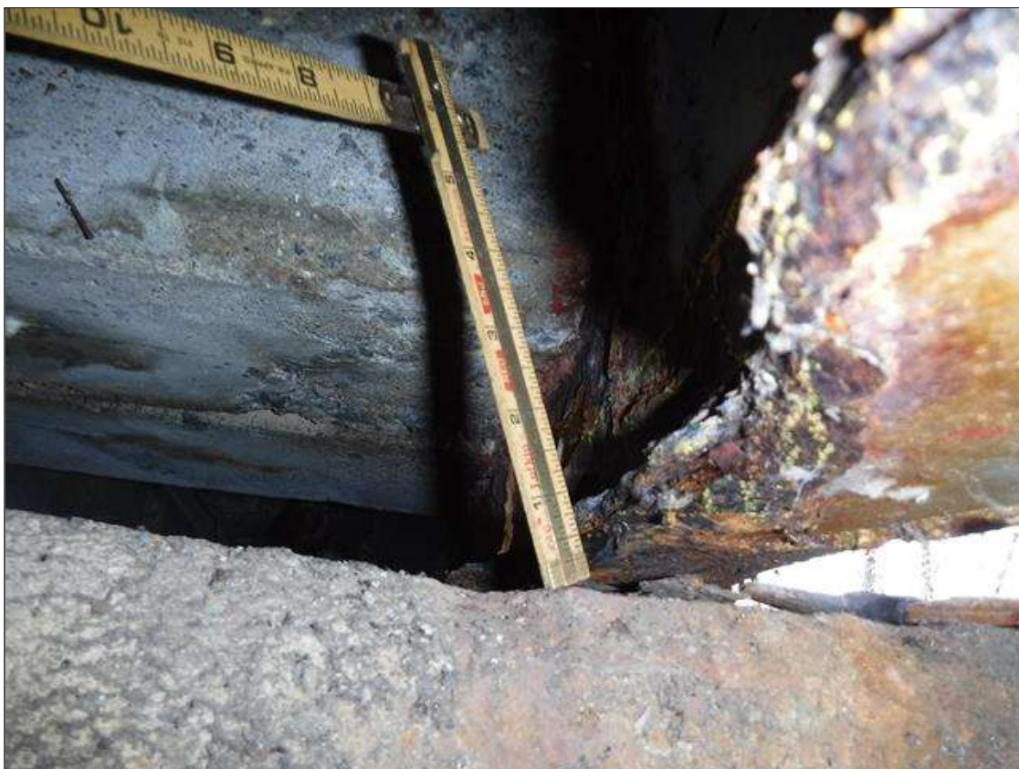
Span 2 Beam 1: 100 % SECTION LOSS BOTTOM FLANGE AT BENT 1 - 1.5 IN WIDE X 14 IN LONG , 5/16 IN REMAINING IN WEB 5 IN HIGH X 1 FOOT LONG PRIORITY MAINTENANCE ISSUED
