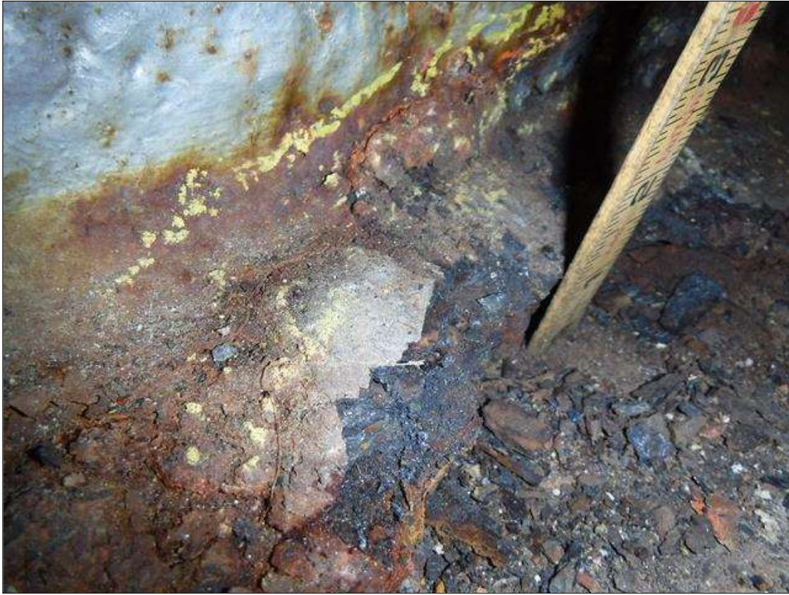
Span 5 Beam 10: SECTION LOSS BOTTOM FLANGE AT BENT 4 IN EDGE 100 % 3/4 IN WIDE X 14 IN LONG , WEB 5/16 IN REMAINING 2 IN HIGH X 8 IN LONG PRIORITY MAINTENANCE ISSUED
