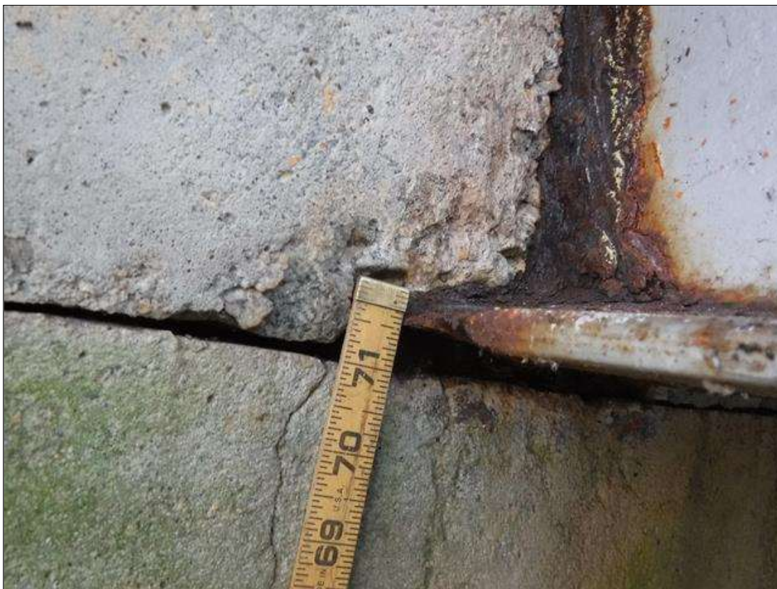
Span 5 Beam 1: SECTION LOSS IN BOTTOM FLANGE AT ABUTMENT 2 - 1/16 IN REMAINING IN EDGE 2 IN LONG , SECTION LOSS WEB 2 IN WIDE 5/16 IN REMAINING PRIORITY MAINTENANCE ISSUED
