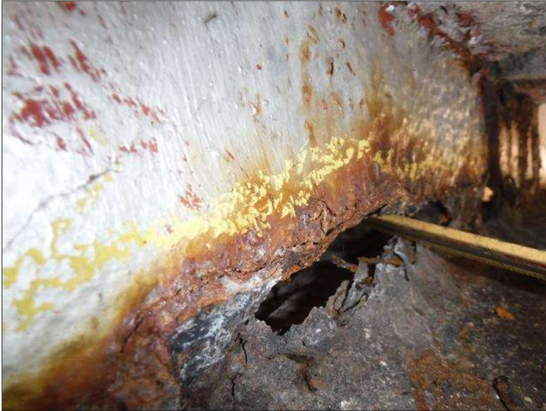
Span 4 Beam 9: SECTION LOSS WEB AT BENT 4 WITH HOLE 1 IN HIGH X 8 IN LONG 1 IN UP FROM BOTTOM FLANGE , SECTION LOSS BOTTOM FLANGE EDGE 100 % 1.5 IN WIDE X 4 IN LONG TAPERING TO FULL REMAINING 2 FOOT LONG PRIORITY MAINTENANCE ISSUED
