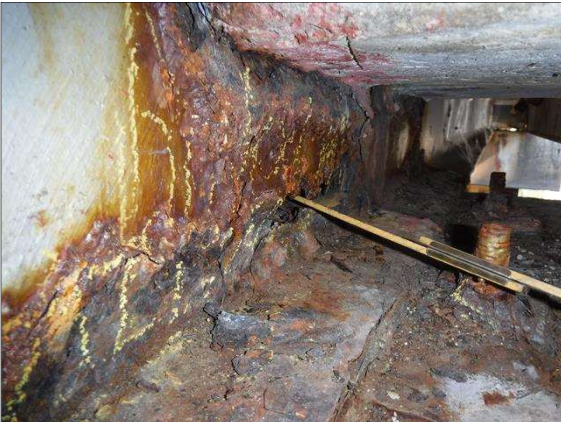
Span 3 Beam 9: SECTION LOSS WEB BENT 3 HOLE 1 IN HIGH X 6 IN LONG 1 IN UP FROM BOTTOM FLANGE, SECTION LOSS 100 % EDGE BOTTOM FLANGE 1 IN WIDE X 14 IN LONG PRIORITY MAINTENANCE ISSUED
