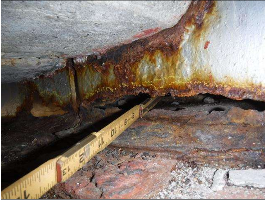
Span 4 Beam 2: SECTION LOSS AT BENT 4 - WEB HAS HOLE 1.5 IN HIGH X 12 IN LONG 1 IN UP FROM BOTTOM FLANGE, 100 % SECTION LOSS EDGE BOTTOM FLANGE 1 IN WIDE 7 IN LONG 5 IN FROM END PRIORITY MAINTENANCE ISSUED
