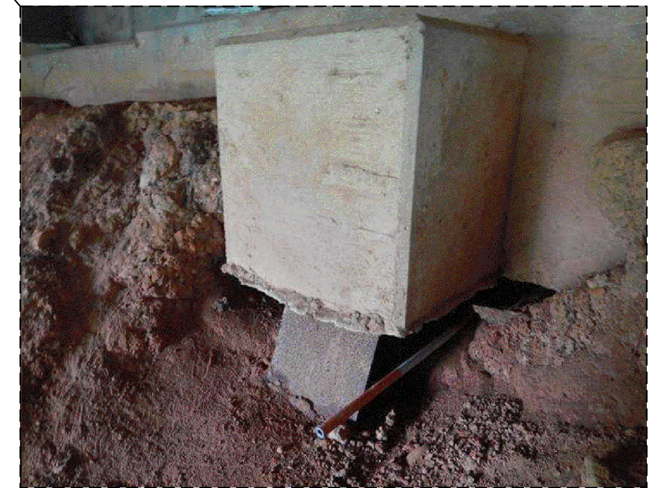
TYPICAL EXPOSED PILE END BENT 1 & 2 SEE SLOPE PROTECTION REPAIR DETAILS FOR LOCATION AND QUANTITIES
