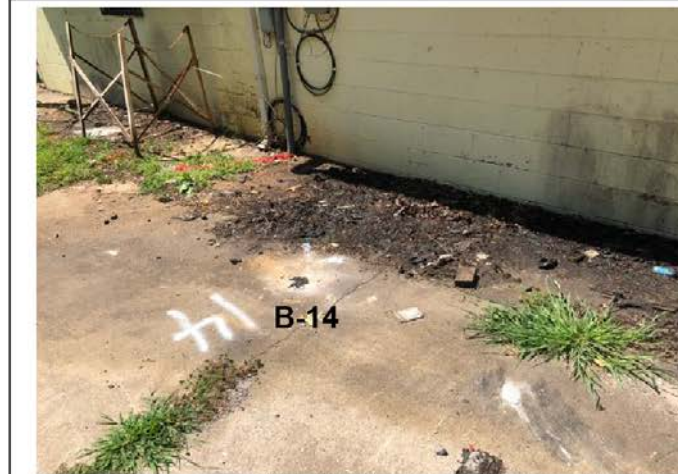
6. Stand for former heating oil AST and stained pavement behind former auto repair facility.
