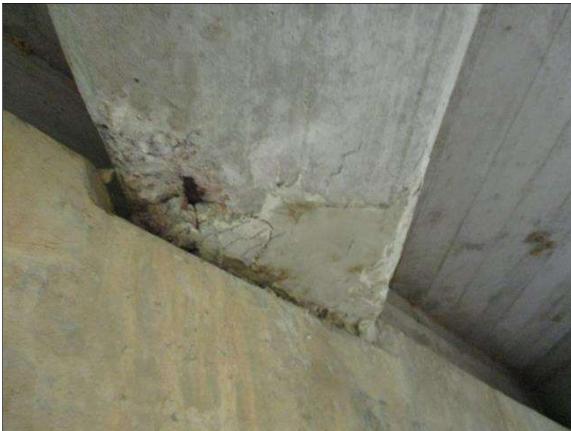
Span 5 Beam 7: SPALL 9" X 9" X 2" DEEP WITH REBAR EXPOSED, AT GIRDER 7 BENT 4 END.
