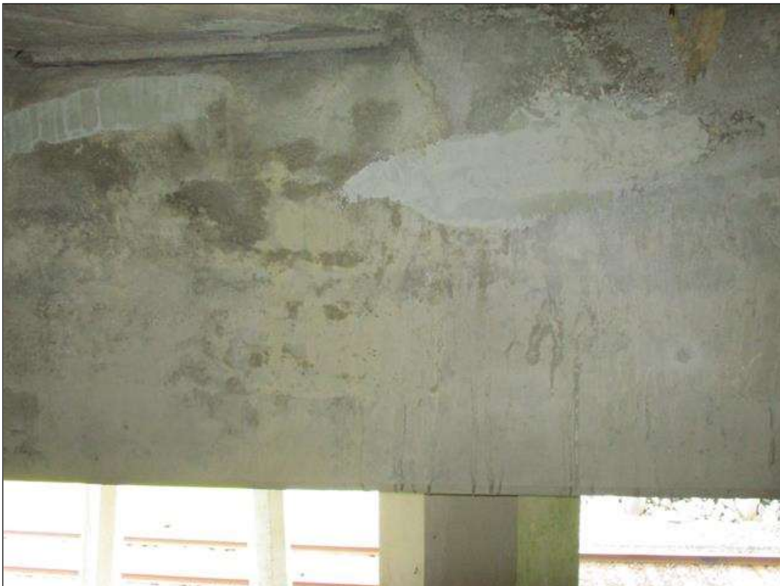
Bent 4 Cap 1: PATCHED AREA 36" WIDE X 14" HIGH UNDER BEAM 6 ON NORTH FACE.
