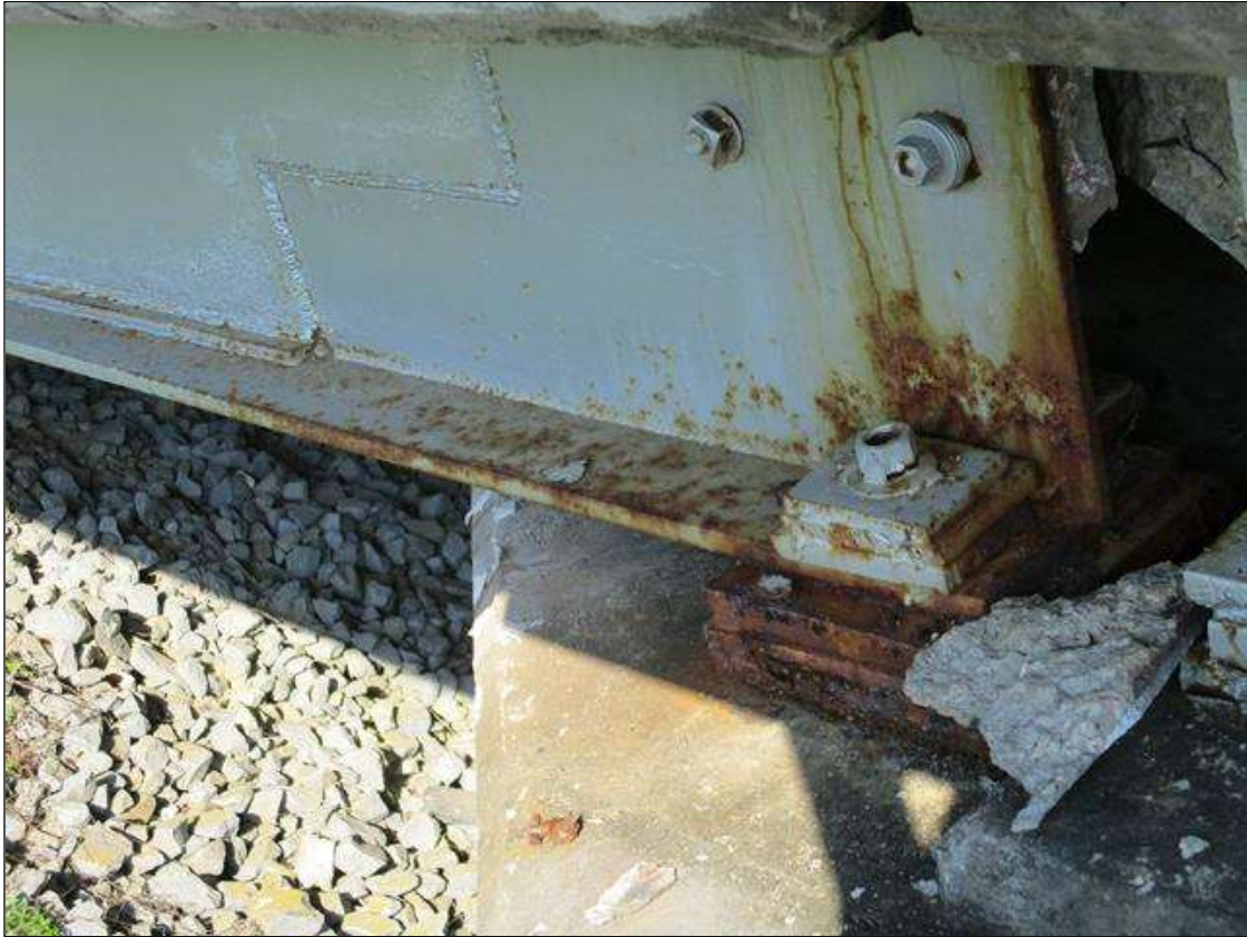
Span 2 Beam 11: FRECKLE SURFACE RUST WITH NO MEASURABLE LOSS OF SECTION ALONG LAST 3' AT BENT 2 END. REPAIR SECTION 24" LONG X 6" IN WEB.
