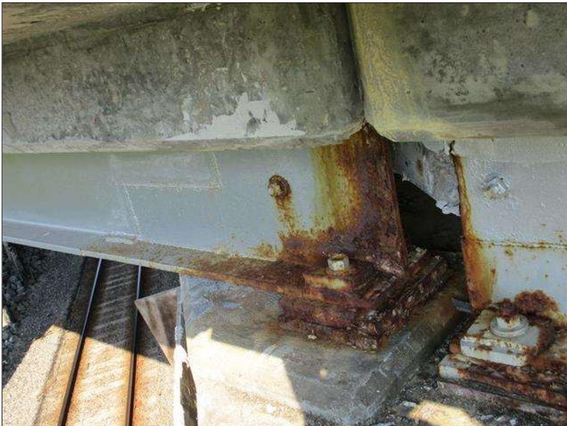
Span 3 Beam 11: FRECKLE SURFACE RUST WITH NO MEASURABLE LOSS OF SECTION ALONG LAST 5' ON WEB AND FLANGES, AT BENT 3 END. REPAIR PLATE SECTION IN WEB 36" LONG X 6" HIGH.
