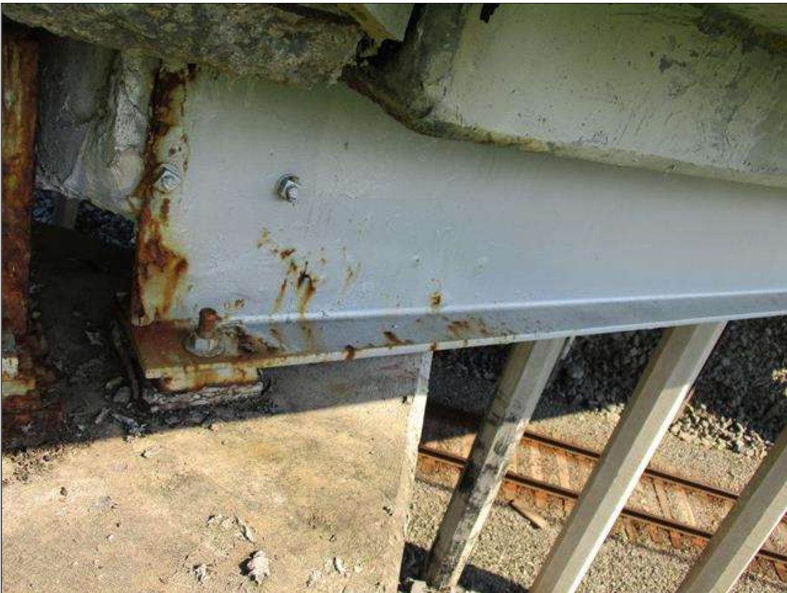
Span 2 Beam 11: FRECKLE SURFACE RUST WITH NO MEASURABLE LOSS OF SECTION ALONG LAST 3' ON WEB AND FLANGES, AT BENT 1 END.
