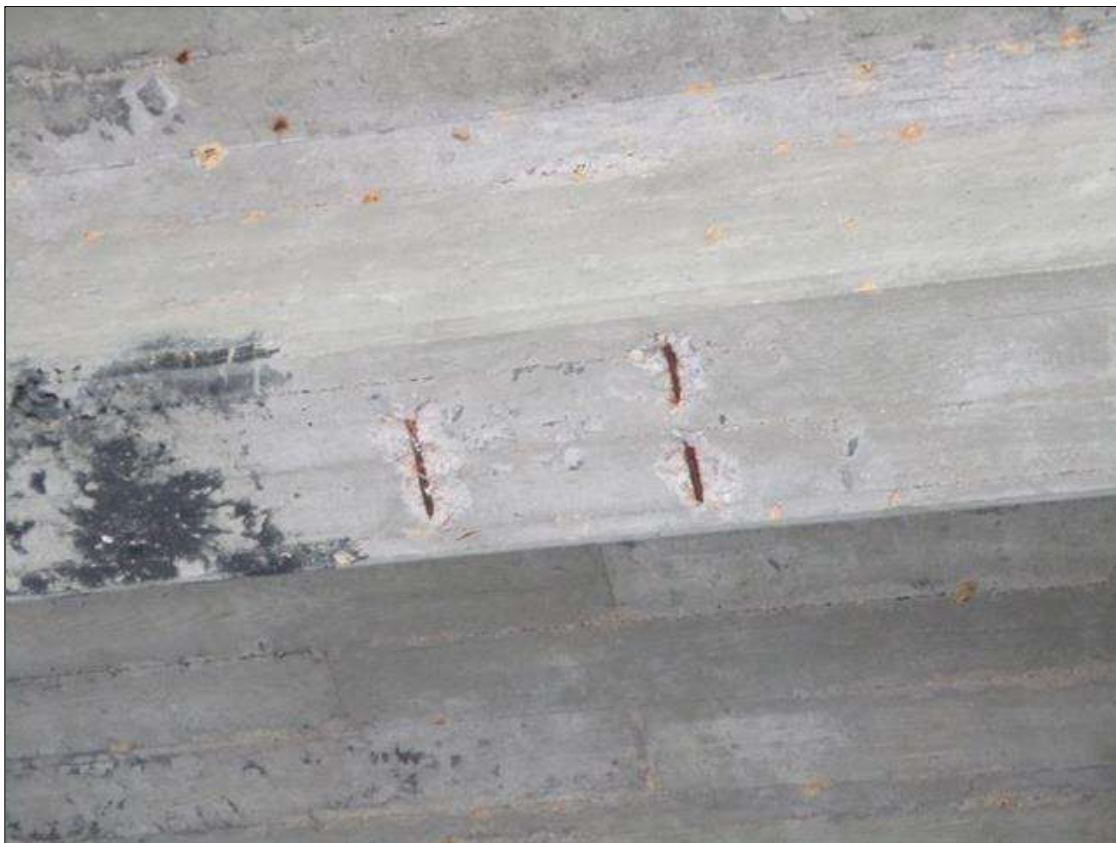
Span 3 Beam 6: SPALLS (3) UP TO 10" WIDE X 4" LONG X 1" DEEP WITH REBAR EXPOSED 8' FROM BENT 2
