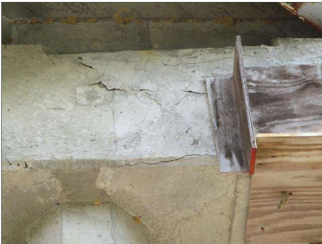
Bent 3 Cap 1: DELAMINATED AREA 4' WIDE X 30" HIGH WITH OLD REPAIR FORMWORK IN PLACE ON SOUTH FACE UNDER BAY 10.
