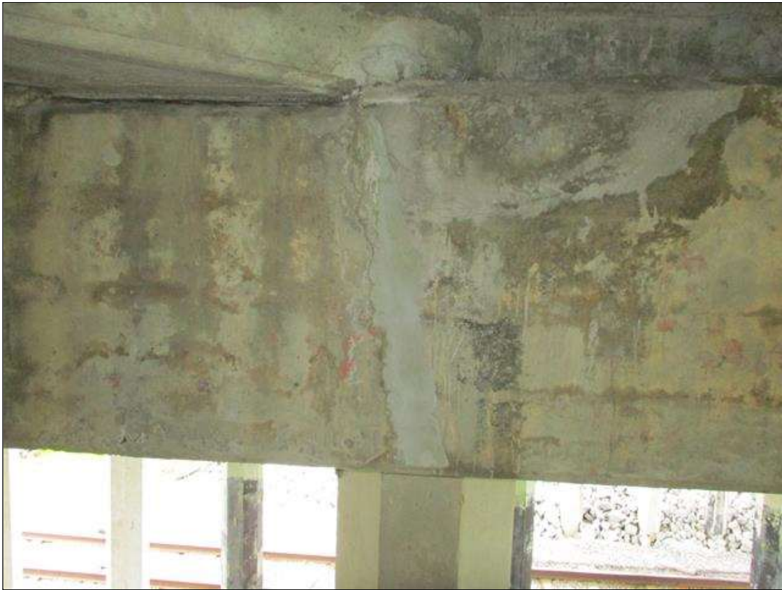
Bent 4 Cap 1: PATCHED AREA 30" WIDE X 14" HIGH AT BEAM 5 ON NORTH FACE.
