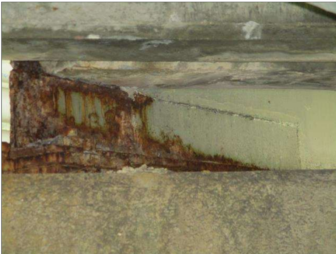
Span 2 Beam 1: FRECKLE SURFACE RUST WITH NO MEASURABLE LOSS OF SECTION ALONG LAST 3' AT BENT 1 END. REPAIR SECTION 30" LONG X 6" HIGH IN WEB AT BENTS 1 AND 2 ENDS.
