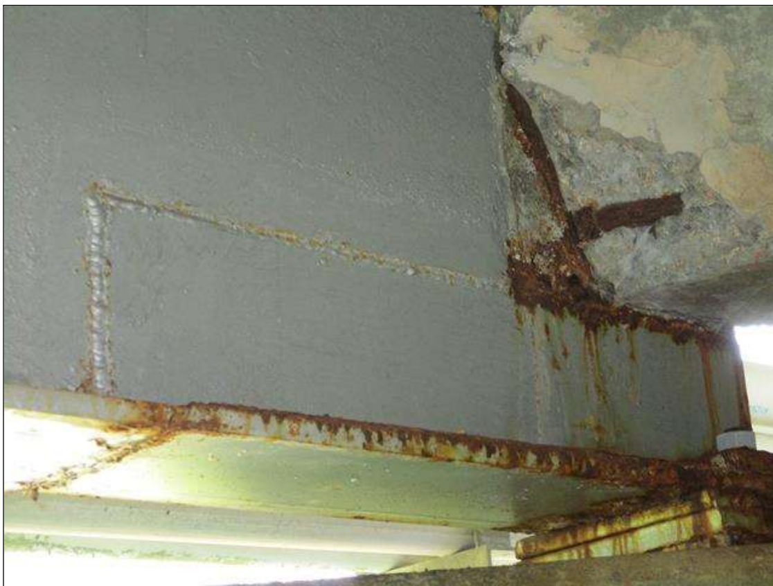
Span 1 Beam 1: FRECKLE SURFACE RUST WITH NO MEASURABLE LOSS OF SECTION ALONG LAST 3' AT BENT 1 END. REPAIR SECTION 30" LONG X 6" HIGH IN WEB AT BENT 1 END.
