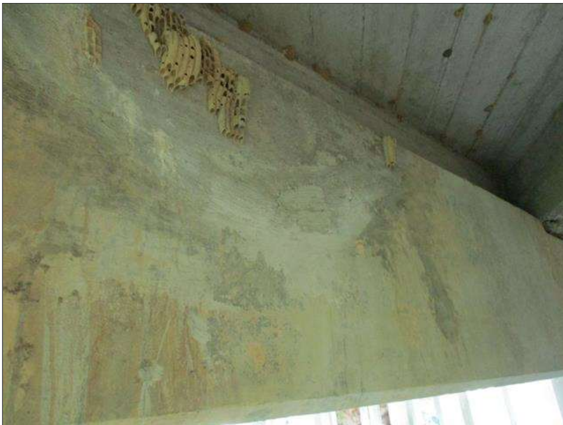
Bent 4 Cap 1: PATCHED AREA 49" WIDE X 17" HIGH BETWEEN GIRDEERS 7 AND 8 ON NORTH FACE.
