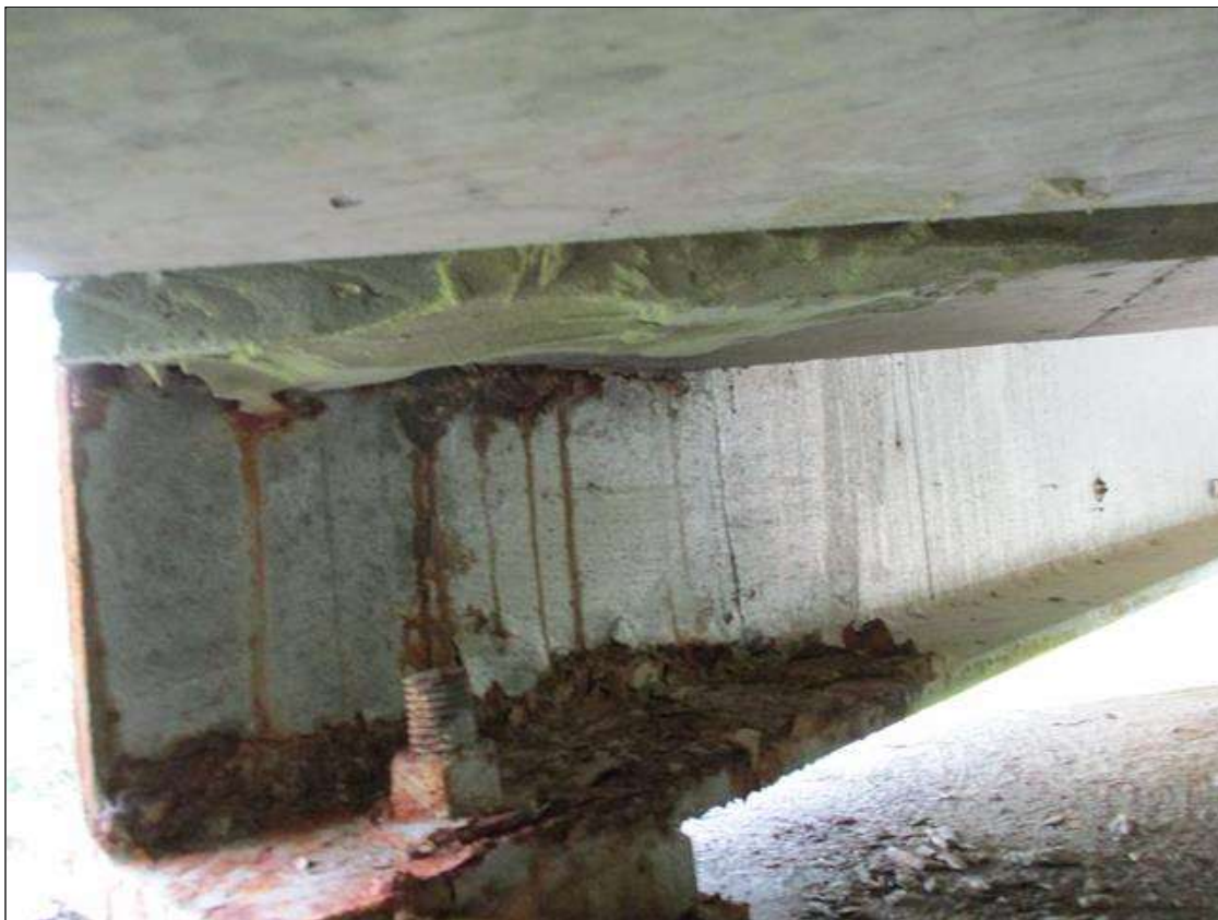
Span 4 Beam 11: LOSS OF SECTION .03" WITH .72" REMAINING BOTTOM FLANGE 9" WIDE X 3' LONG AT BENT 4 END.
