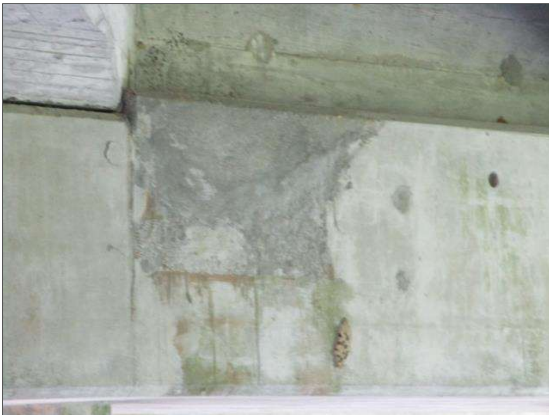
Bent 2 Cap 1: PATCHED AREA 30" WIDE X 18" HIGH UNDER BEAM 7 ON SOUTH FACE.
