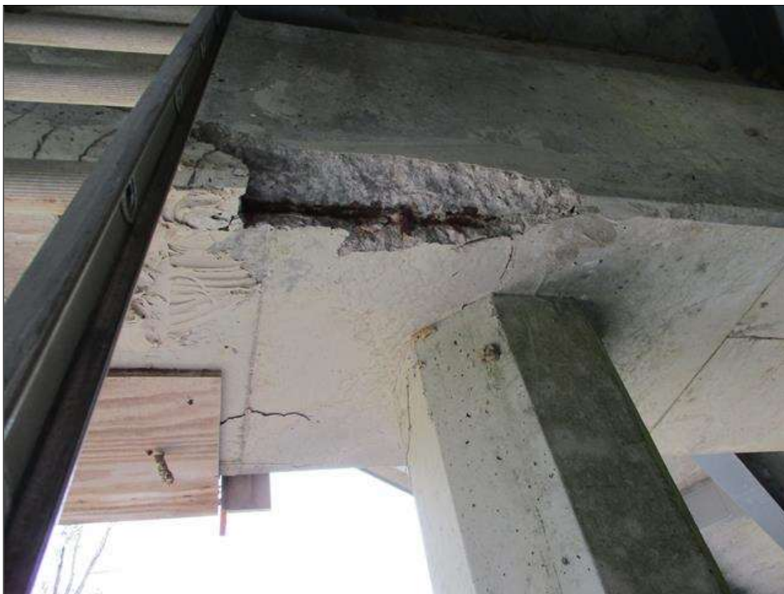
Bent 3 Cap 1: SPALL 30" WIDE X 10" HIGH X 3-1/2" DEEP BETWEEN PILES 10 AND 11 ON NORTH FACE. (PRIORITY MAINTENANCE)
