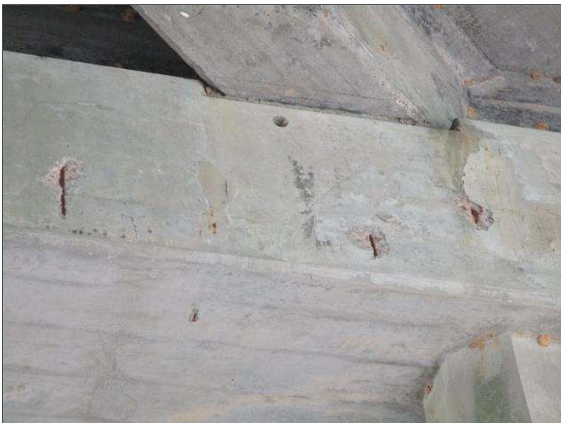
Bent 2 Cap 1: SPALLS (3) (2) 6" X 6" X 1/2" DEEP AND 11" WIDE X 5" LONG X 3/4" DEEP WITH REBAR EXPOSED OVER PILE 6.
