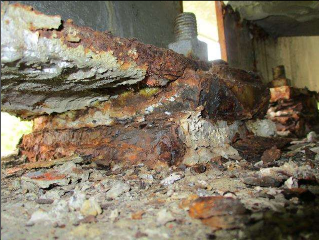
Span 5 Beam 11 Near Bearing: SPAN 5 BEAM. 11 N/B: LOSS OF SECTION .063" ALONG PLATE EDGES WITH PACK RUST BETWEEN PLATES.
