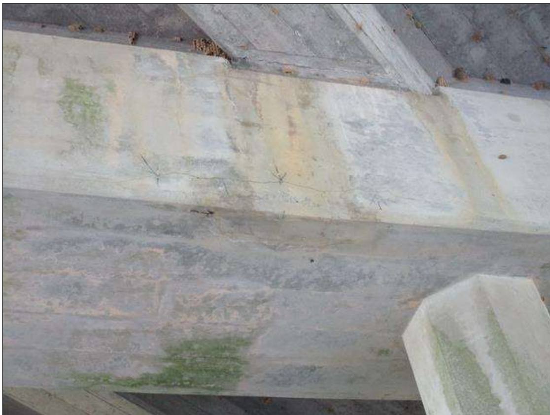
Bent 1 Cap 1: HORIZONTAL CRACK UP TO .03" OPEN 3' LONG UNDER BEAM 7 ON NORTH FACE.
