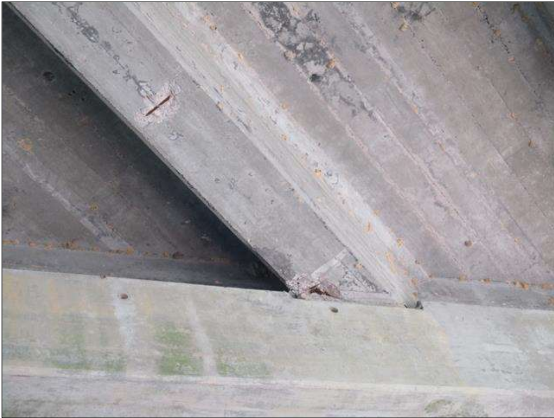
Span 3 Beam 6: SPALLS (2) 10" WIDE X 8" LONG X 3/4" DEEP REBAR EXPOSED , 6' FROM BENT 3 END AND 7" WIDE X 12" LONG X 1" DEEP AT BENT 3 END.
