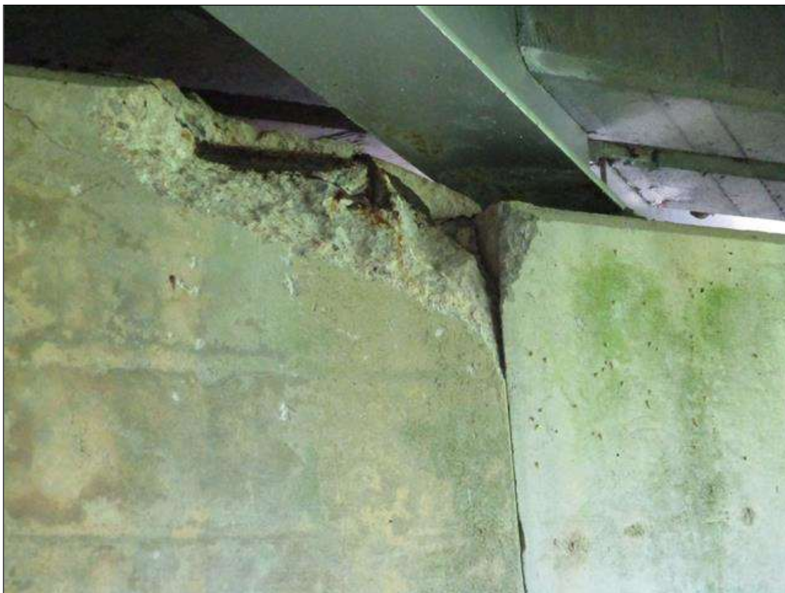
Bent 1 Cap 1: SPALL 24" WIDE X 12" HIGH X 4" DEEP WITH 10% LOSS OF SECTION AT EXPOSED REBAR UNDER BEAM 9 SOUTH FACE. (PRIORITY MAINTENANCE)
