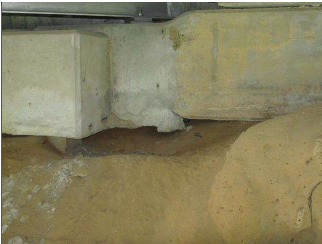
NORTH EARTH SLOPE UNDERMINING UNDER CAP AT BEAM 3: 9" HIGH VERTICAL X 6' WIDE X 26" DEEP (LATERAL).
