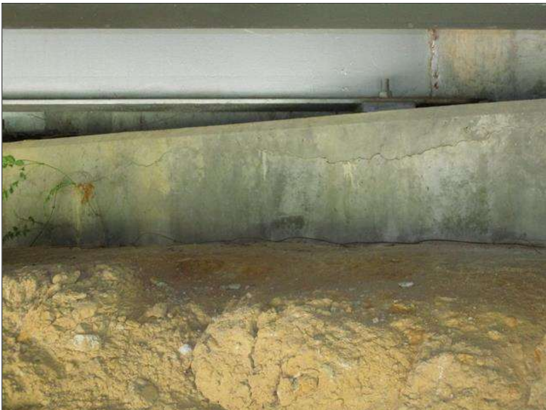
Bent 1 Cap 1: HORIZONTAL CRACKING .063" OPEN UNDER BEAMS 9 AND 10.
