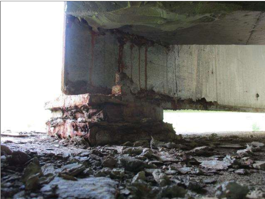
Span 4 Beam 11 Near Bearing: SPAN 4 BEAM. 11 F/B: LOSS OF SECTION .063" ALONG PLATE EDGES WITH PACK RUST BETWEEN PLATES.
