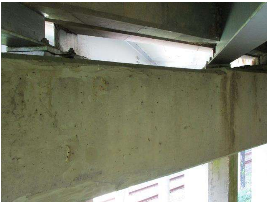
Bent 4 Cap 1: HORIZONTAL CRACKING UP TO .063" OPEN 3' LONG BETWEEN BEAMS 9 AND 10 ON NORTH FACE.
