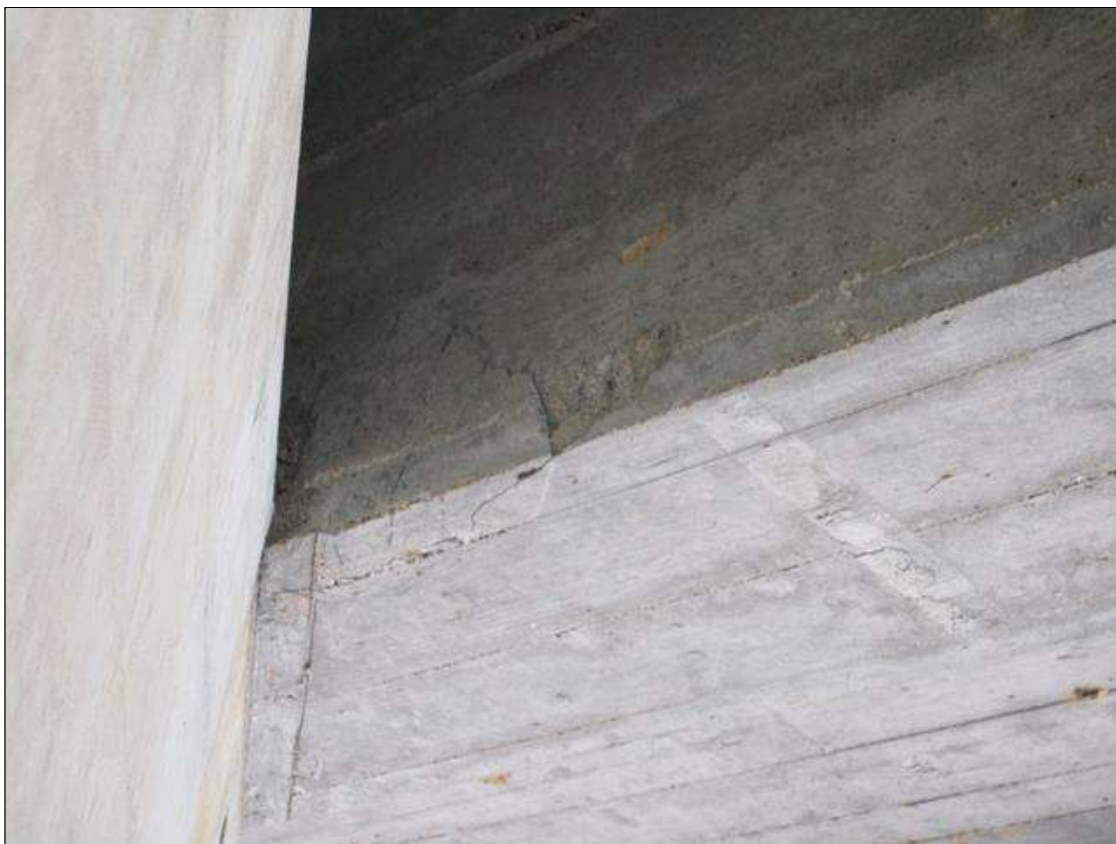
Span 4 Beam 6: DELAMINATED AREA 4" WIDE X 18" LONG WITH .063" SEPARATION, BOTTOM LEFT FACE AT BENT 4 END.
