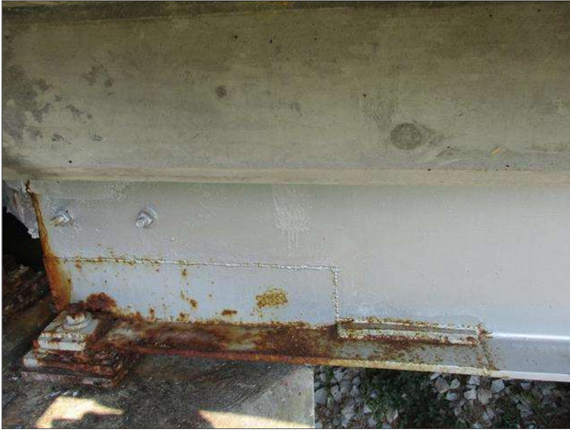
Span 4 Beam 11: FRECKLE SURFACE RUST WITH WEB REPAIR PLATE 36" LONG X 6" HIGH AT BENT 4 END.
