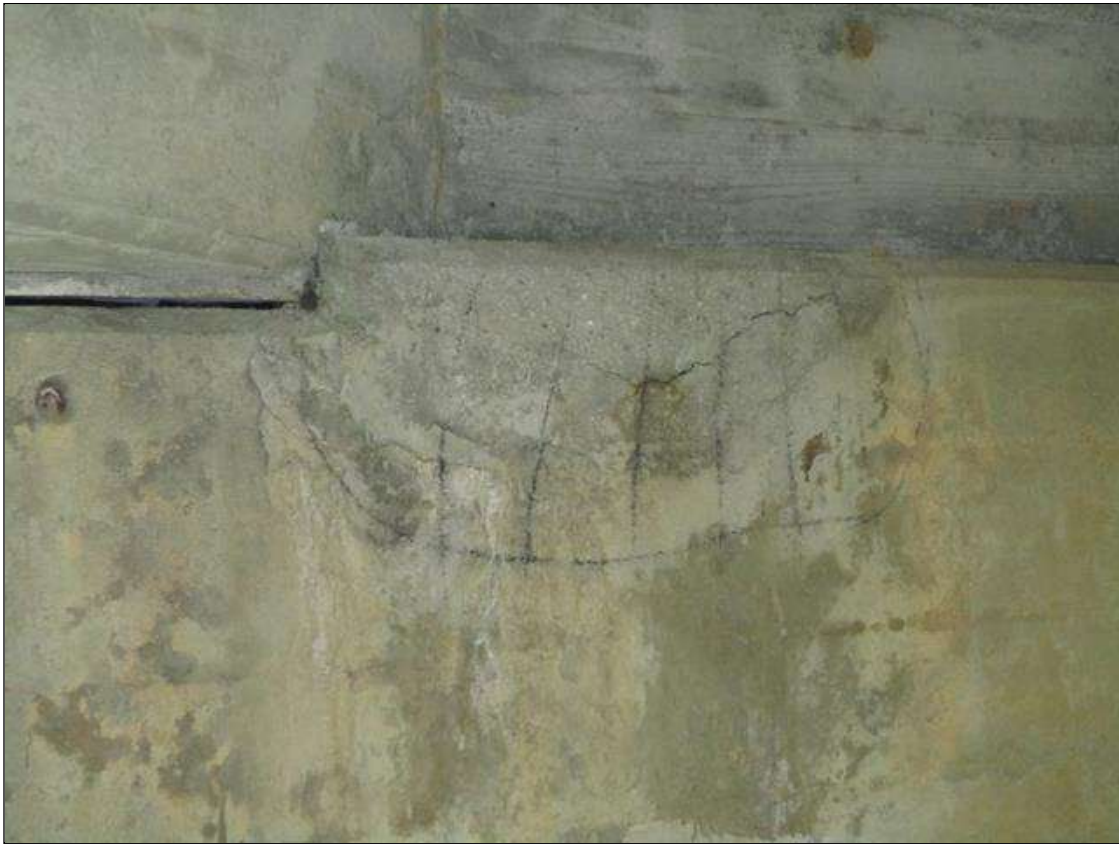
Bent 1 Cap 1: DELAMINATED AREA 36" WIDE X 19" HIGH WITH .125" SEPARATION UNDER BEAM 5 ON SOUTH FACE.
