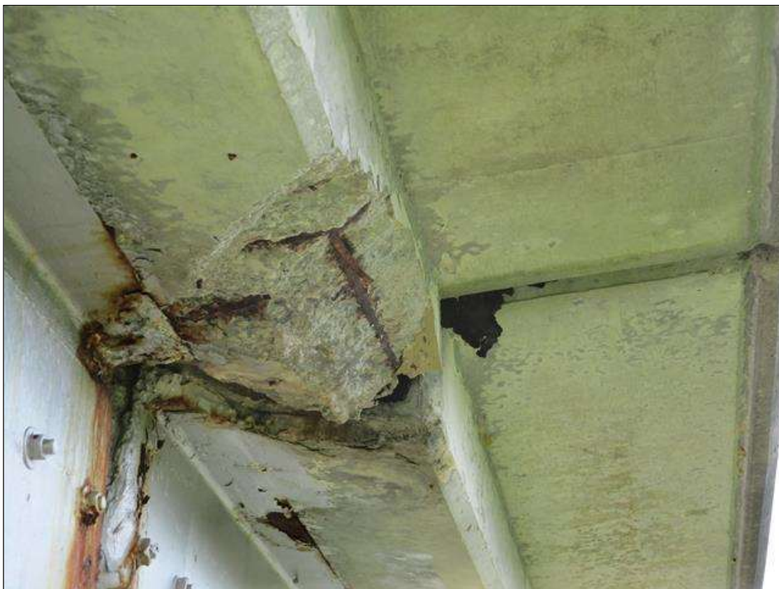
Span 1 Deck: SPALL 24" LONG X 18" WIDE X 4" DEEP WITH 10% LOSS OF SECTION ON EXPOSED REBAR AT BENT 1 END OVERHANG. (PRIORITY MAINTENANCE)
