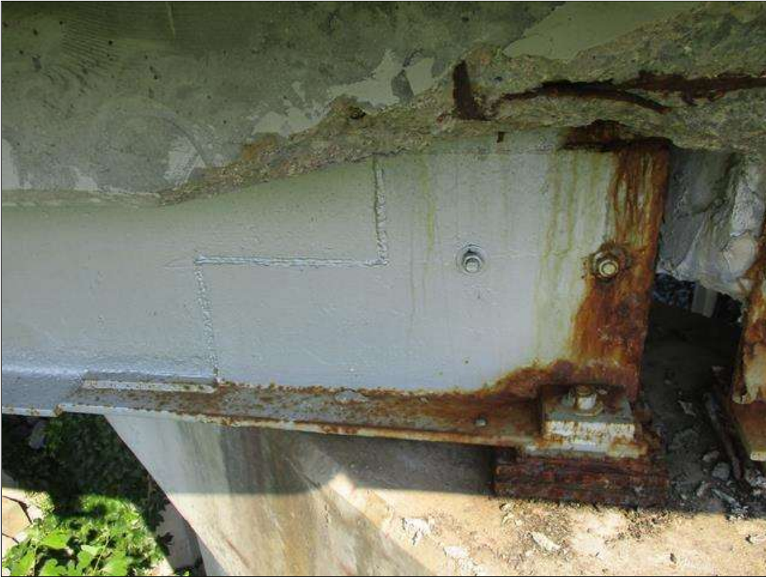
Span 1 Beam 11: FRECKLE SURFACE RUST WITH NO MEASURABLE LOSS OF SECTION ALONG LAST 3' AT BENT 1 END. REPAIR SECTION 30" LONG X 18" HIGH IN WEB AT BENT 1 END.
