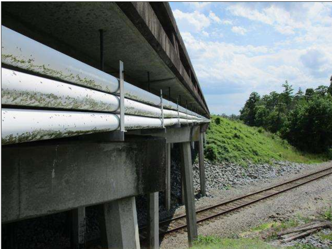
UTILITY LEFT SIDE 6- 4" PVC PIPES.
