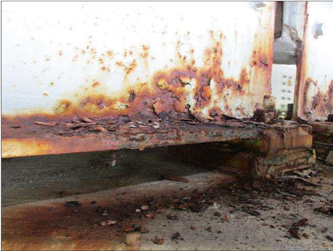
Span 4 Beam 1: FRECKLE SURFACE RUST WITH NO MEASURABLE LOSS OF SECTION ON BOTTOM FLANGE 9" WIDE X 3' LONG AND BOTTOM 3" HIGH OF WEB AT BENT 4 END.
