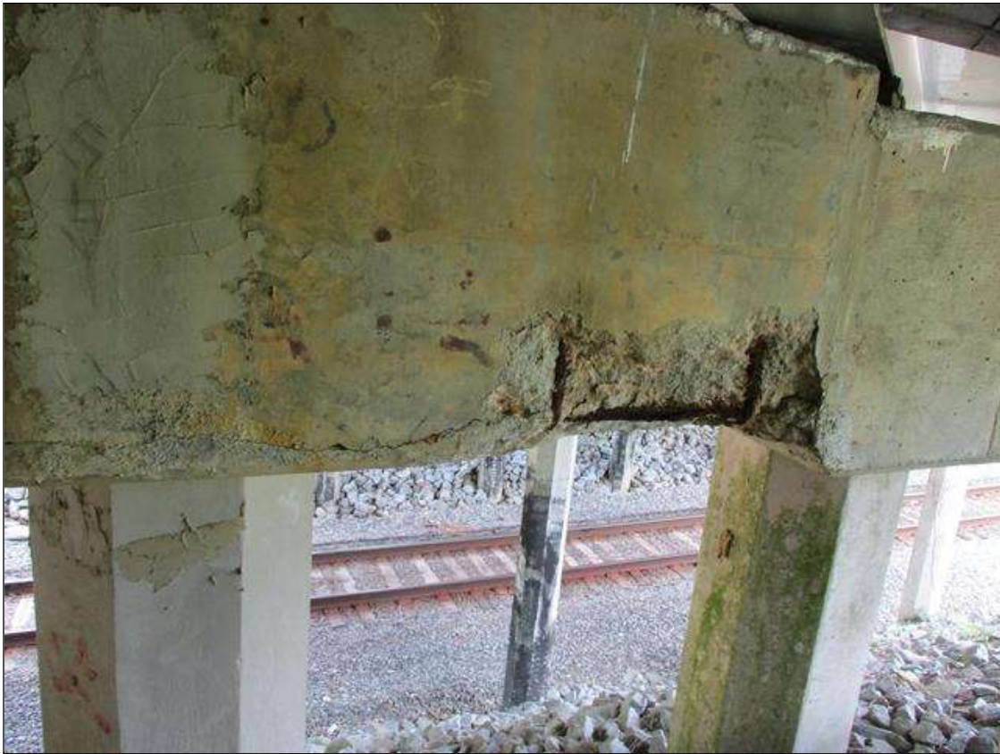
Bent 4 Cap 1: SPALL 28" WIDE X 18" HIGH X 4" DEEP WITH 10% LOSS OF SECTION AT EXPOSED REBAR BETWEEN PILES 3 AND 4 ON NORTH FACE. HORIZONTAL CRACK .04" OPEN EXTENDING FROM SPALL 3' LONG. (PRIORITY MAINTENANCE)
