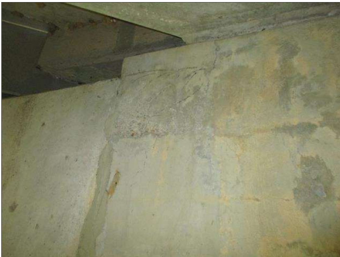
Bent 4 Cap 1: DELAMINATED AREA 11" WIDE X 24" HIGH WITH .125" SEPARATION UNDER BEAM 8 ON NORTH FACE.
