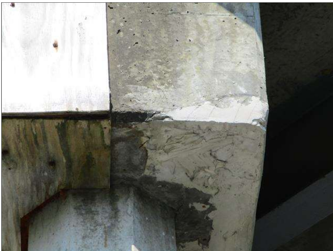
Bent 3 Cap 1: DELAMINATED AREA 12" WIDE X 6" HIGH ON RIGHT END.
