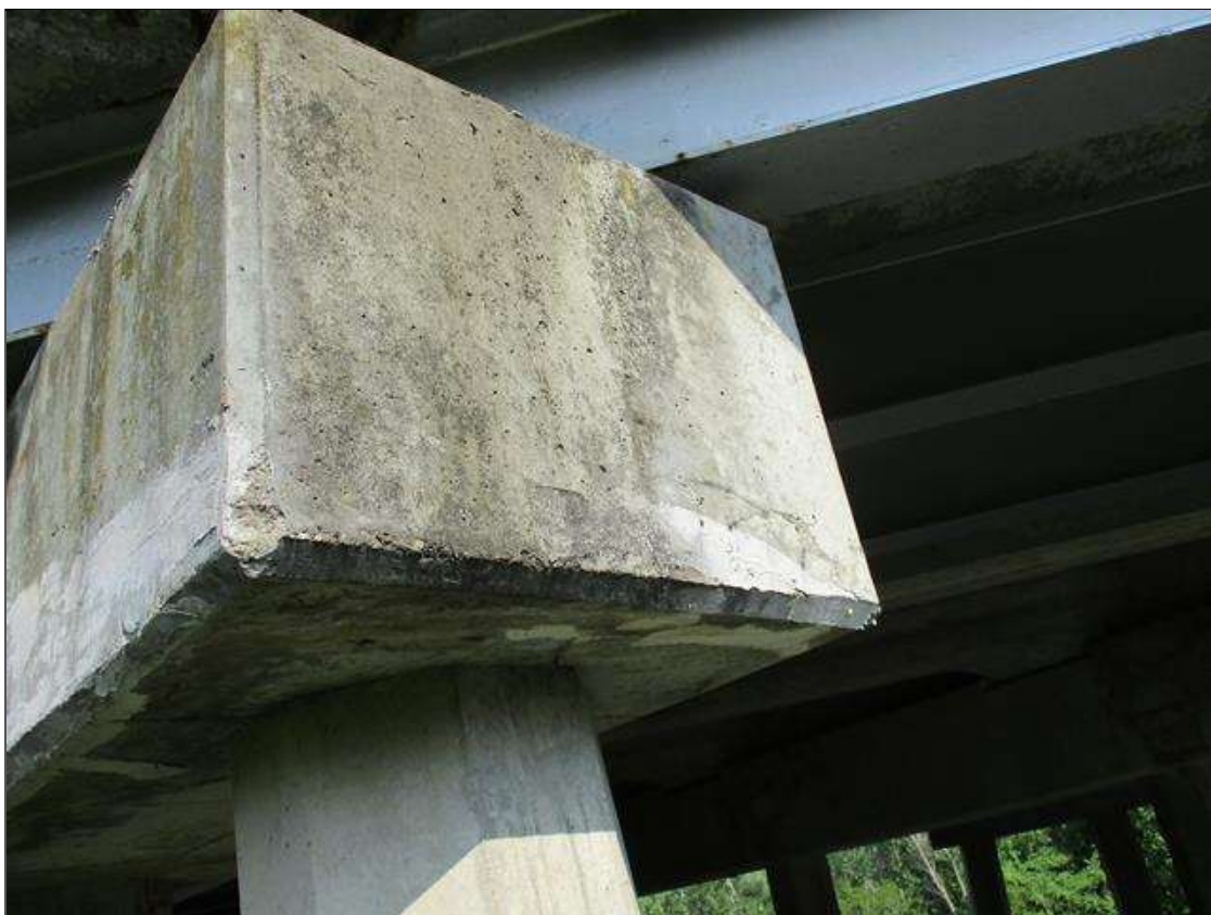
Bent 1 Cap 1: DELAMINATED AREA 24" WIDE X 7" HIGH ON RIGHT END.
