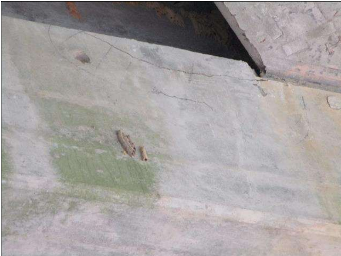
Bent 3 Cap 1: DELAMINATED AREA 36" WIDE X 16" HIGH WITH .063" SEPARATION UNDER BEAM 7 ON SOUTH FACE.
