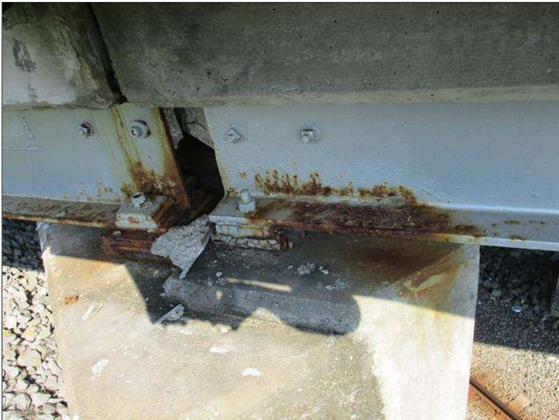
Span 3 Beam 11: FRECKLE SURFACE RUST WITH NO MEASURABLE LOSS OF SECTION ALONG BEGINNING 5' ON WEB AND FLANGES, AT BENT 2 END.
