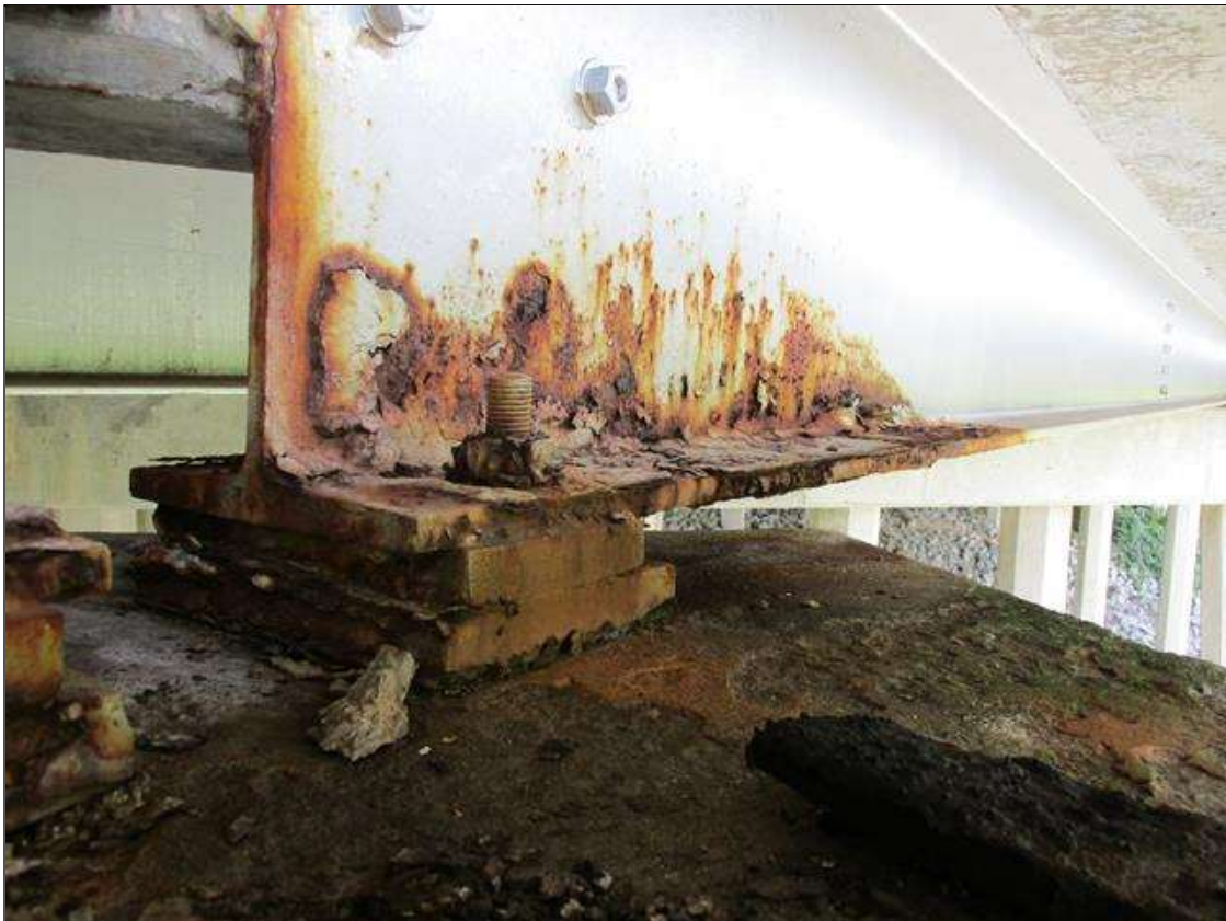
Span 5 Beam 1: FRECKLE SURFACE RUST WITH NO MEASURABLE LOSS OF SECTION ON BOTTOM FLANGE 9" WIDE X 3' LONG AND BOTTOM 3" HIGH OF WEB AT BENT 4 END.
