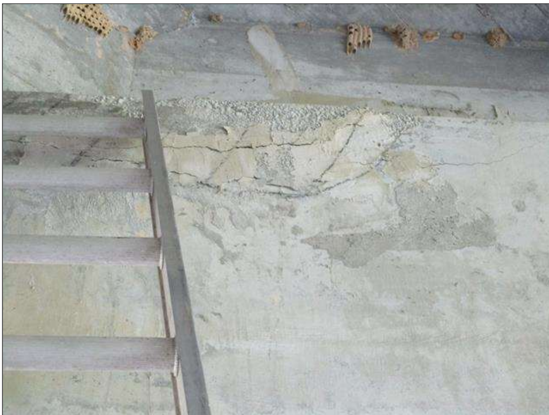
Bent 3 Cap 1: DELAMINATED AREA 33" WIDE X 13" HIGH WITH .125" SEPARATION UNDER BEAM 6 ON NORTH FACE.
