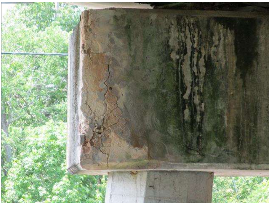
Bent 2 Cap 1: PATCHWORK ON LEFT END HAS MAP CRACKING 063" OPEN AND DELAMINATED 10" WIDE X 24" HIGH.
