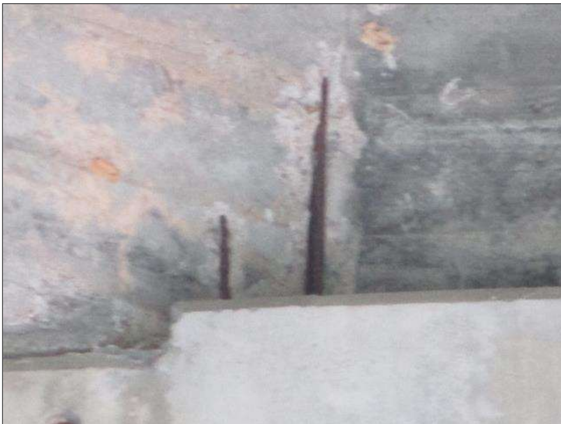
Span 3 Beam 5: SPALLS (2) 6" X 6" AND 6" WIDE X 14" HIGH BOTH 1/2" DEEP REBAR EXPOSED AT RIGHT SIDE, BENT 3 END.
