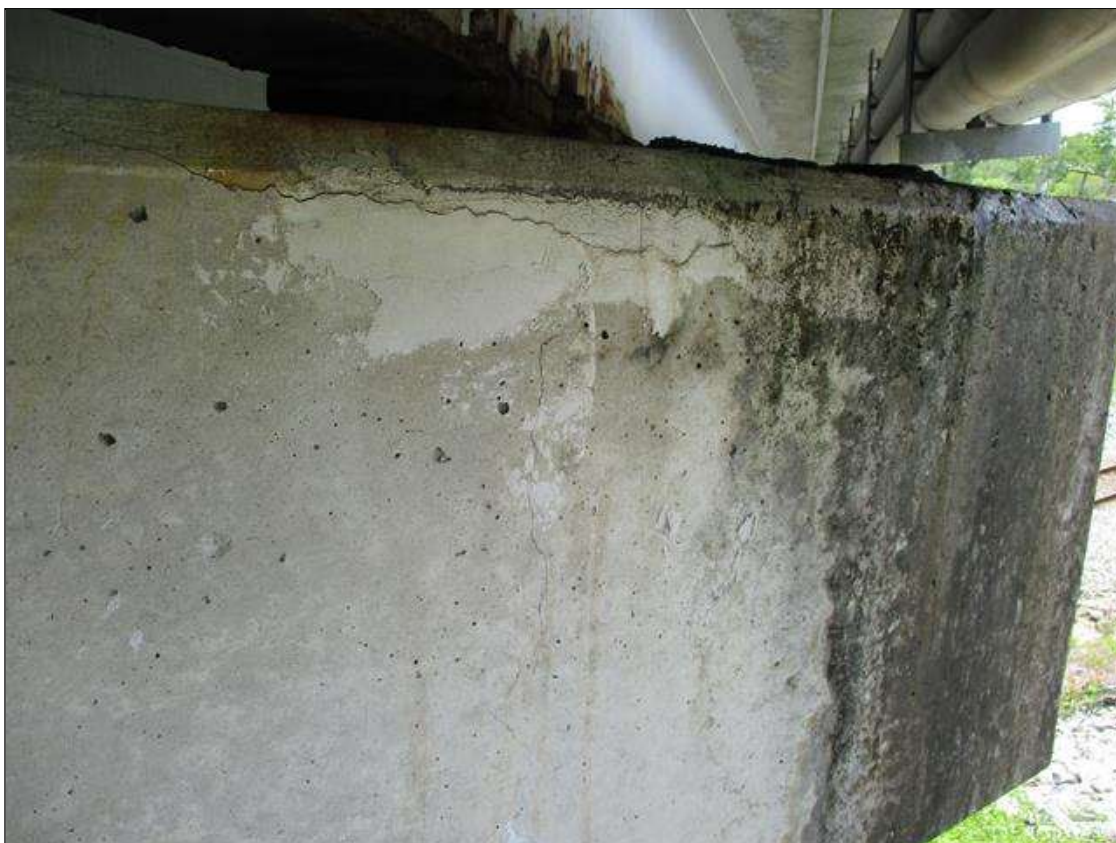
Bent 4 Cap 1: HORIZONTAL CRACKING .03" OPEN 2' LONG UNDER BEAM 1 ON NORTH FACE.
