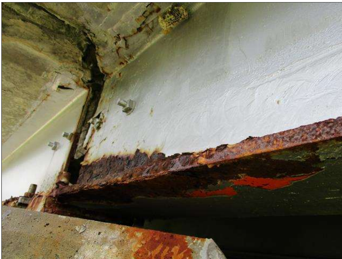
Span 5 Beam 11: LOSS OF SECTION .03" WITH .72" REMAINING BOTTOM FLANGE 9" WIDE X 3' LONG AT BENT 4 END.
