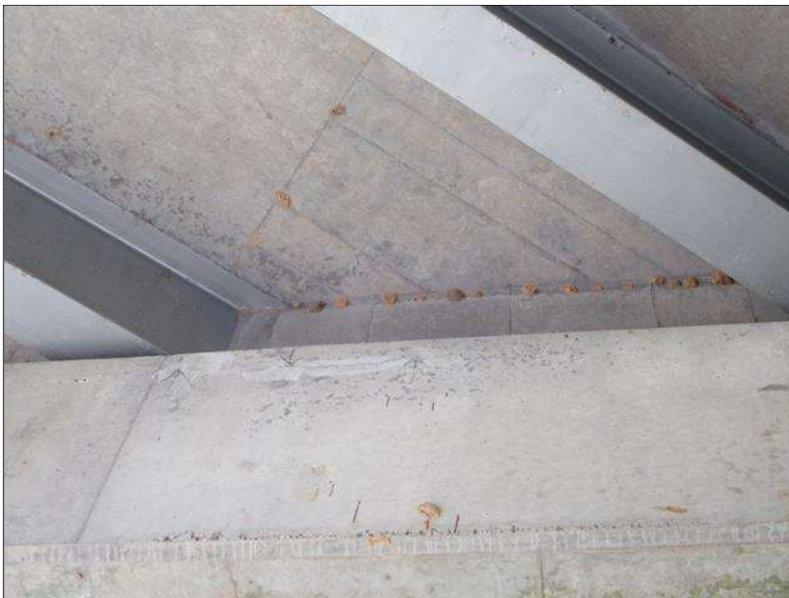
Bent 1 Cap 1: HORIZONTAL CRACKING .03" OPEN 3' LONG UNDER BEAM 10 ON NORTH FACE.
