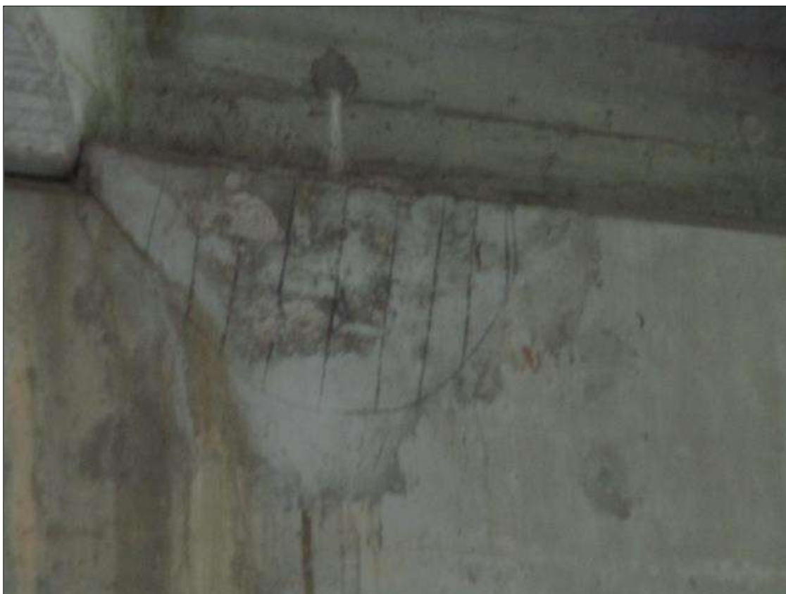
Bent 2 Cap 1: DELAMINATED PATCH 33" WIDE X 20" HIGH UNDER BEAM 6 ON SOUTH FACE.
