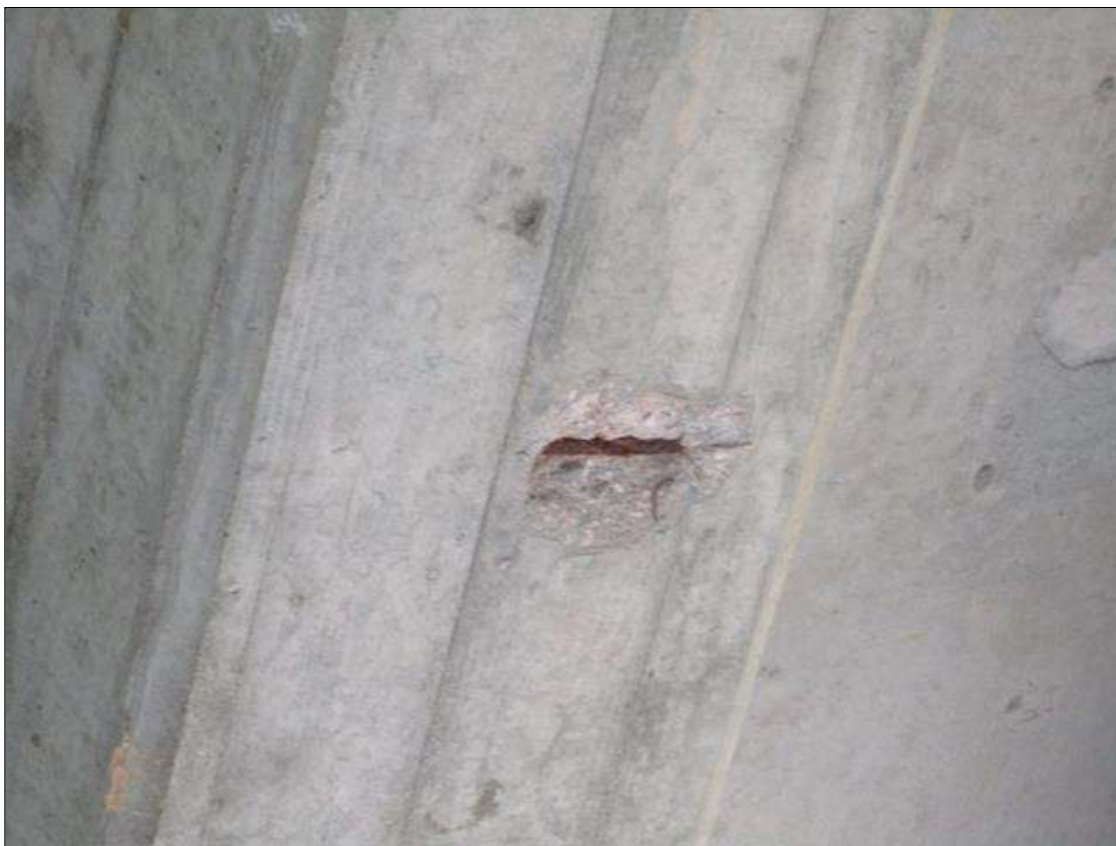
Span 2 Beam 8: SPALL 7" X 7" X 3/4" DEEP REBAR EXPOSED BOTTOM FACE, 8' FROM BENT 1 END
