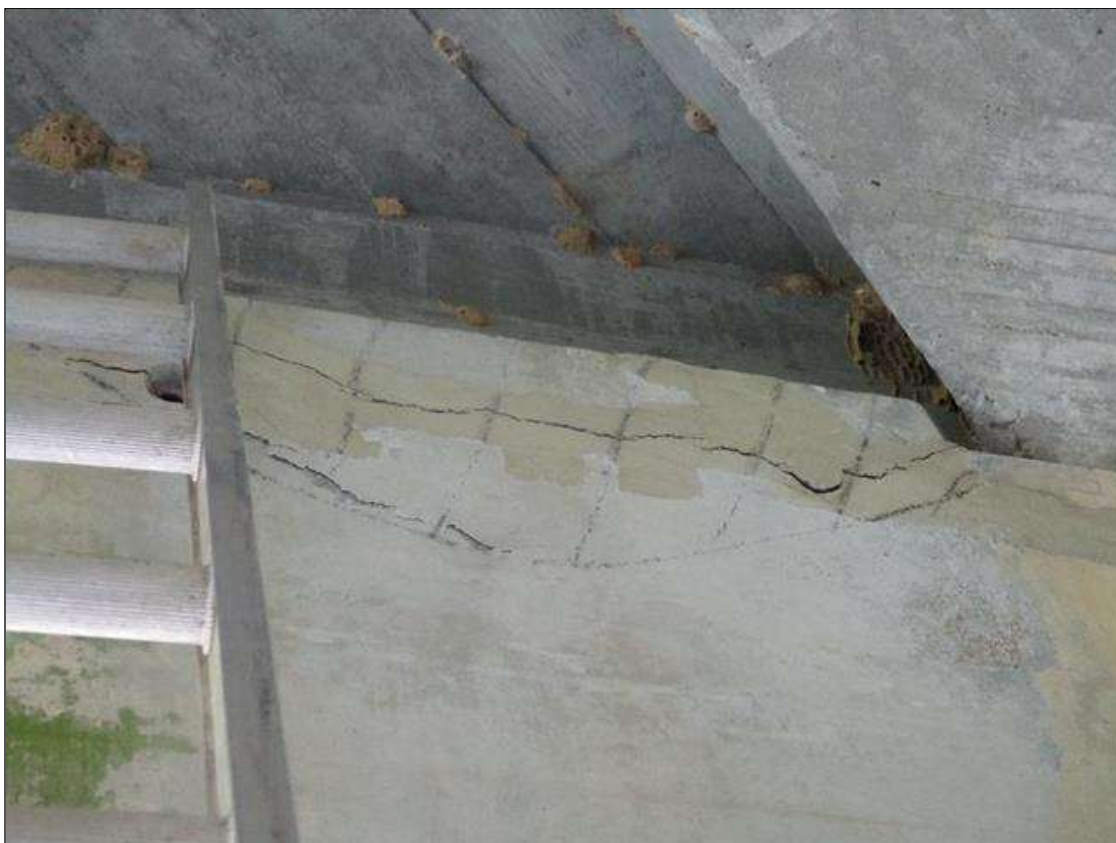
Bent 3 Cap 1: DELAMINATED AREA 45" WIDE X 18" HIGH WITH .125" SEPARATION UNDER BEAM 7 ON NORTH FACE.
