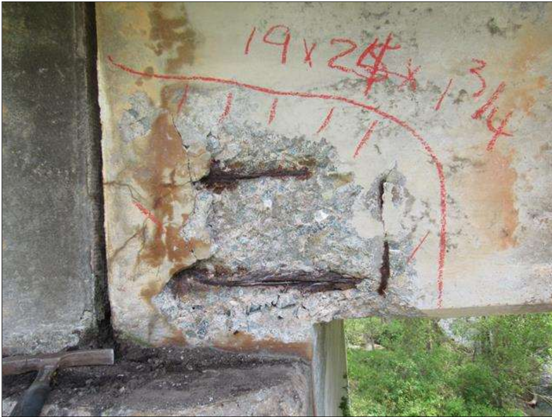
Span 2 Beam 5: 2 Feet of Delamination/Spall/Patched Area: Spall greater than 1 in. deep or greater than 6 in. diameter. Patched area that is unsound or showing distress. Does not warrant structural review. SPAN 2 RIGHT SIDE OF GIRDER 5 HAS A CRACKED SPALL DELAMINATED AREA OVER BENT 1 19" HIGH FM END OUT 24" 1 3/4" DEEP WITH REBAR AND STIRRUPS EXPOSED.
