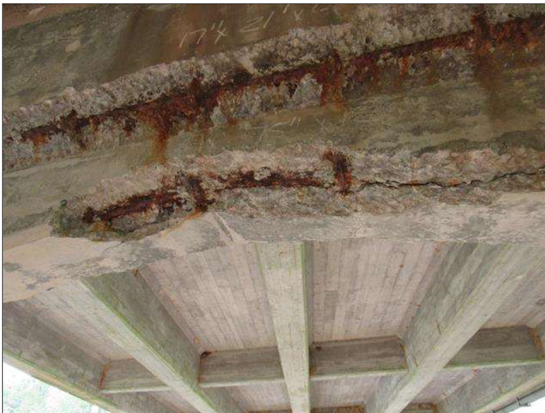
BENT 4 EAST FACE AND BOTTOM OF HUANCH UNDER G3 CRACKED SPALL AND DELAMINATED 9" WIDE 75" LONG 6" UNDER BOTTOM WITH REBAR AND STIRRUPS EXPOSED.
