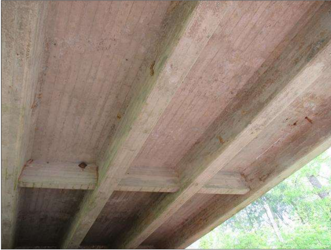
Span 5 Deck: 1400 Square Feet of Cracking (RC and Other): Width 0.012-0.05 in. or spacing of 1.0-3.0 ft. SPAN 5 BOTTOM OF DECK HAS SCATTERED MAP CRACKING WITH EFFLO STAINS.
