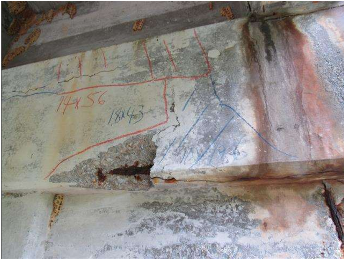
BENT 1 EAST OF CAP HAS CRACKED SPALL DELAM AREA ALONG BOTTOM OF CAP RIGHT SIDE OF G1 18" UP FACE 43" LONG SPALL IS 10" X 19" X 6" WITH LARGE REBAR EXP
