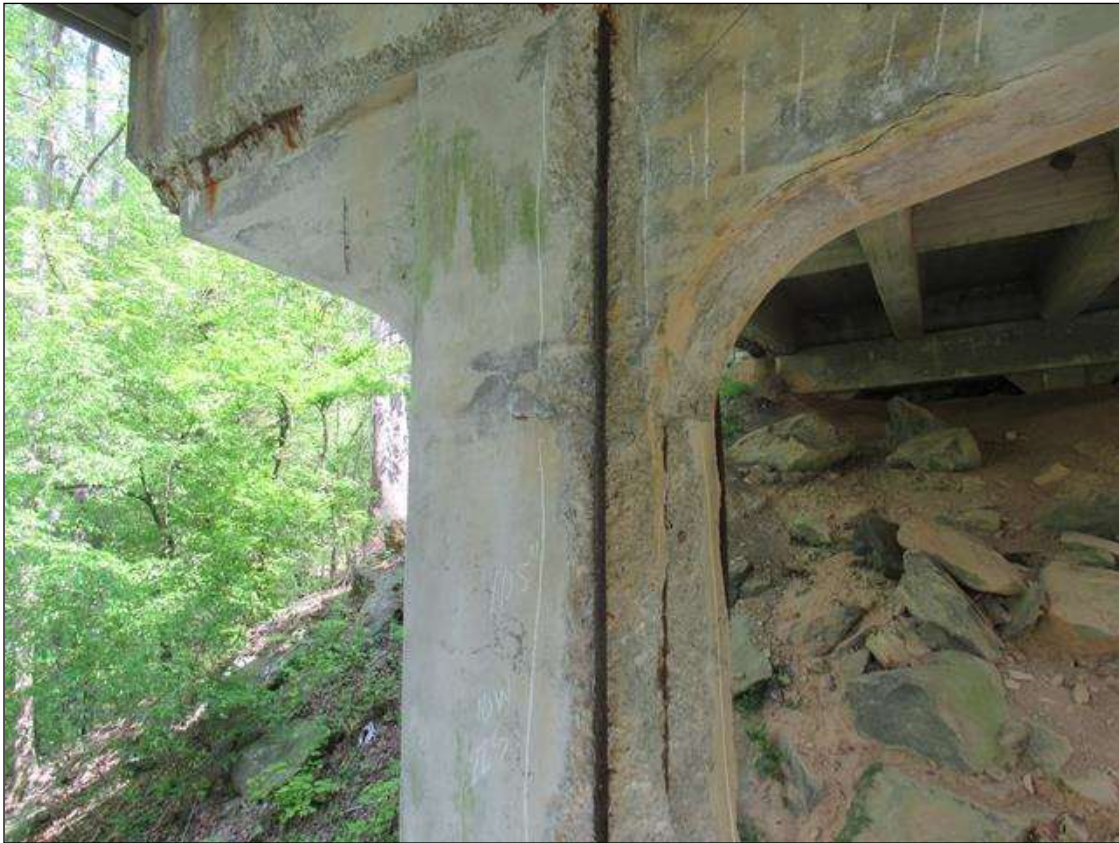
BENT 4 PILE 1 CRACKED SPALL DELAMINATED AREA ON SW CORNER OF PILE BOTTOM CAP DOWN 105" 22" ON SOUTH FACE AND 10" ON WEST REBAR EXPOSED.
