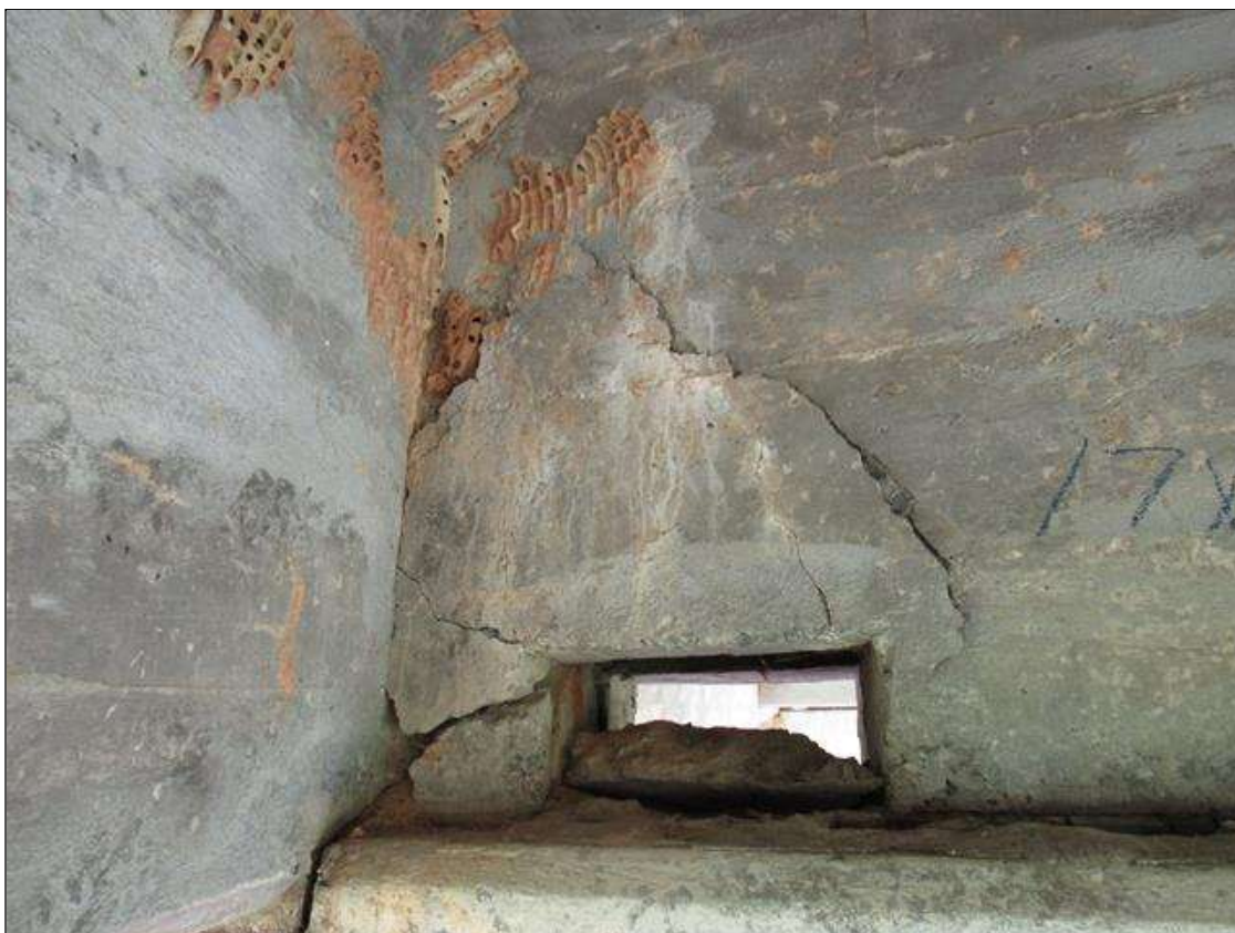
END DIAPHRAGM IN BAY 3 IS CRACKED AND DELAMINATED RIGHT SIDE OF GIRDER 3. 17" X 20".
