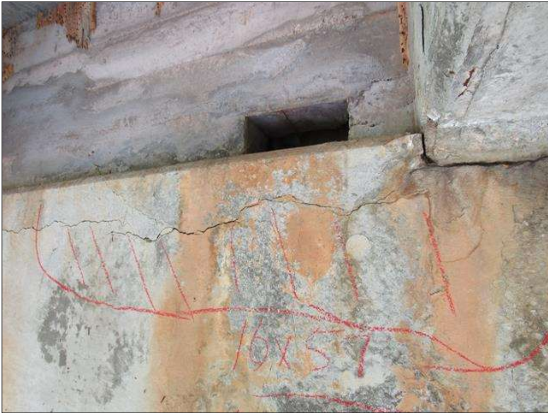
Bent 1 Cap : 0 Feet of Delamination/Spall/Patched Area: Delaminated. Spall 1 inch or less deep or 6 inches or less in diameter. Patched area that is sound BENT 1 EAST FACE OF CAP HAS A CRACKED DELAMINATED AREA ALONG THE TOP RIGHT SIDE OF GIRDER 3. 16" DOWN FACE 57" LONG.
