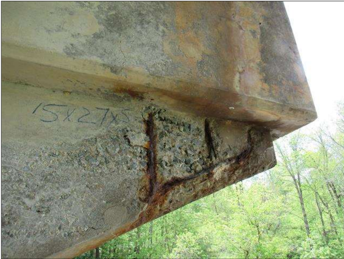
BENT 2 WEST FACE OF HAUNCH AREA UNDER G 5 CRACKED SPALL AND DELAMIN. 15" DOWN THE FACE 27" LONG AND 5" UNDER BOTTOM WITH REBAR AND STIRRUPS EXPOSED.
