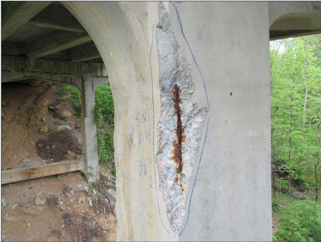
BENT 3 NW CORNER OF PILE 1 SPALL AREA 33" BELOW CAP EXTENDS DOWN 38". 5" ON NORTH 10" ON WEST WITH LARGE REBAR EXPOSED.
