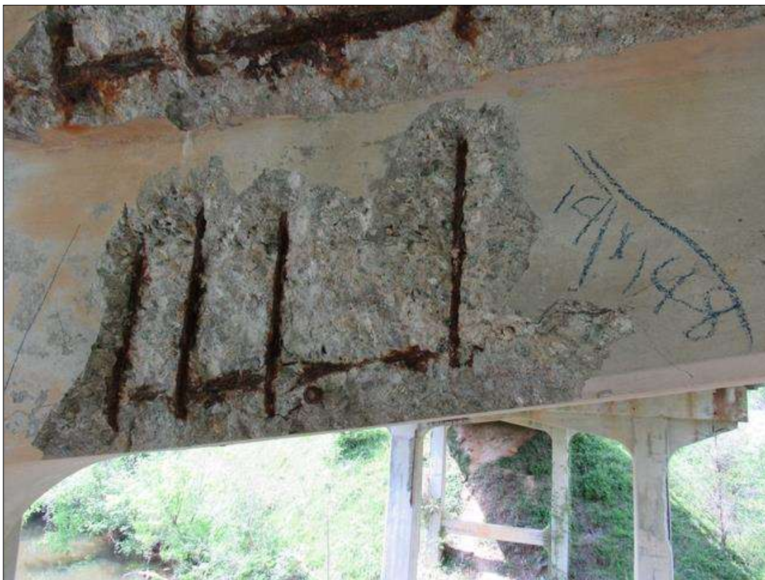
BENT 3 EAST FACE OF HAUNCH UNDER BOTTOM OF CAP SPALL DELAMINATED 19" HIGH 48" LONG 2" DEEP WITH REBAR AND STIRRUPS EXPOSED.
