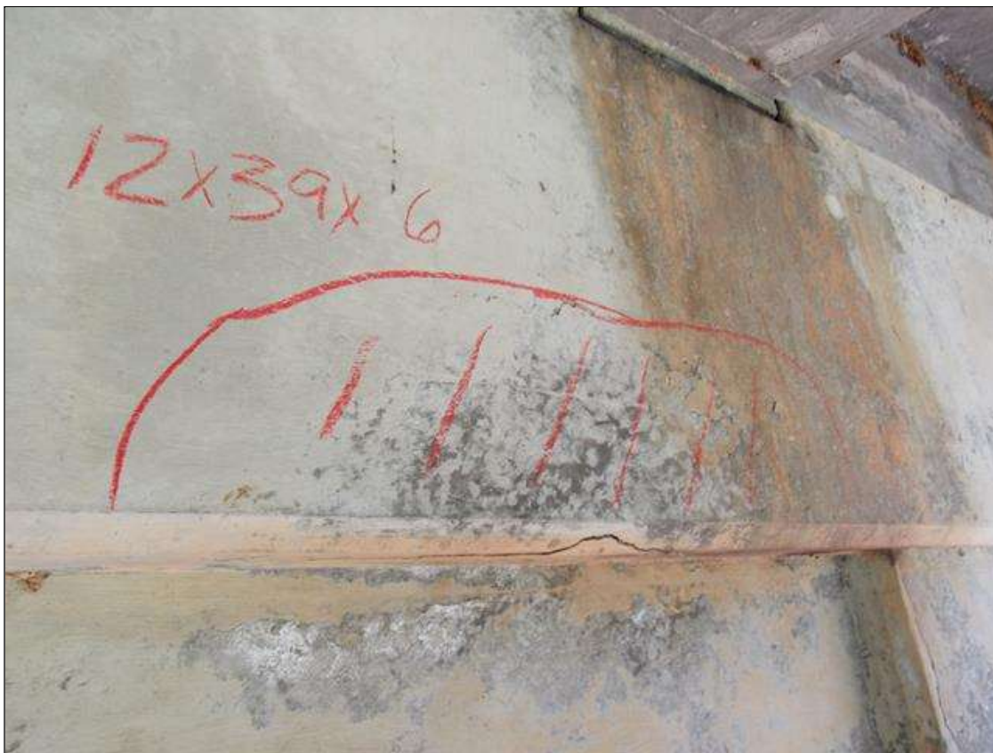
Bent 2 Cap : 4 Feet of Delamination/Spall/Patched Area: Delaminated. Spall 1 inch or less deep or 6 inches or less in diameter. Patched area that is sound BENT 2 WEST FACE OF CAP CRACKED AND DELAMINATED AREA UNDER BOTTOM EDGE 12" UP FACE 39" LONG 6" UNDER BOTTOM.
