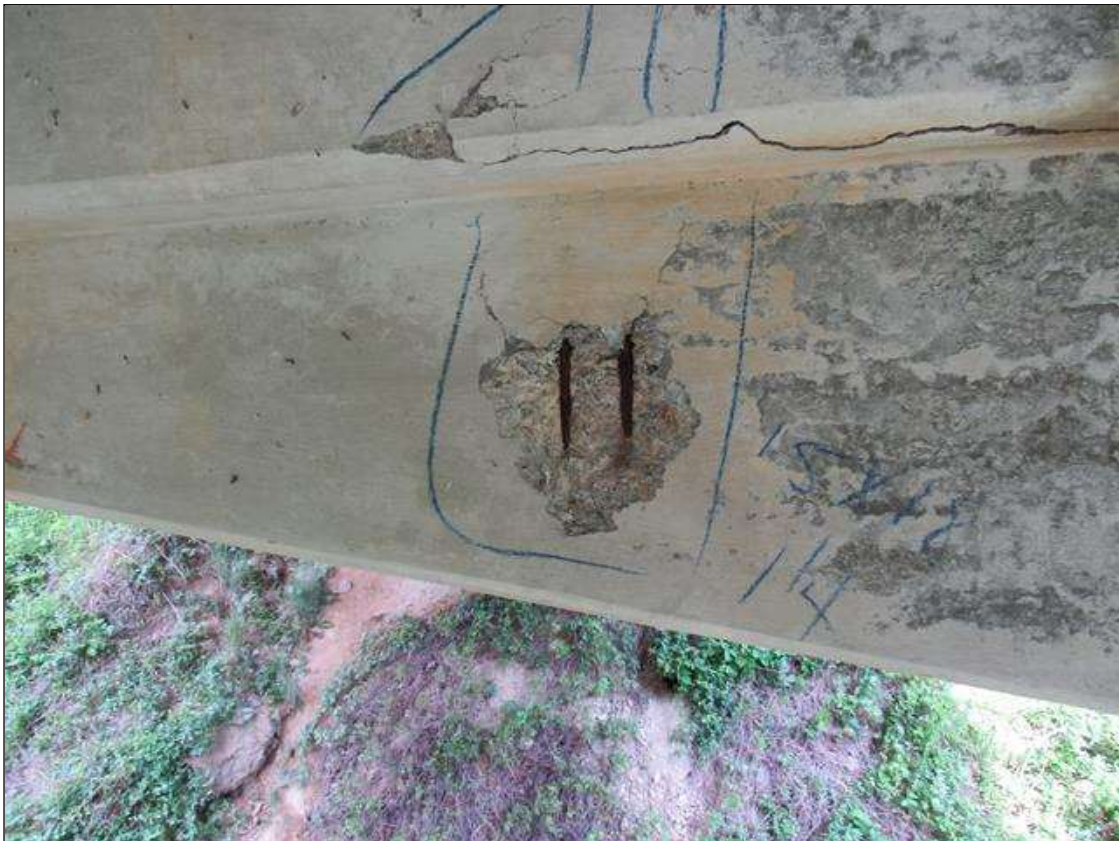
HAUNCH AREA UNDER BENT 1 CAP HAS A CRACKED SPALL DELAMINATED AREA 3' TO RIGHT OF PILE 1 15" X 18" X 1 1/4" DEEP WITH VERTICAL REBAR EXPOSED.
