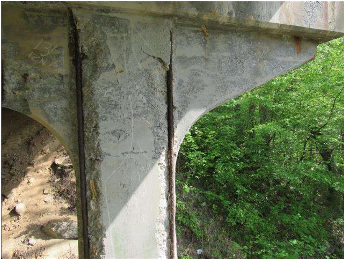
Bent 4 Pile 2: 0 Each of Delamination/Spall/Patched Area: Spall greater than 1 in. deep or greater than 6 in. diameter. Patched area that is unsound or showing distress. Does not warrant structural review. BENT 4 PILE 2 CRACKED DELAMINATED SPALL AREA SW CORNER OF PILE FM BOTTOM OF CAP DOWN 93". 8" ON WEST FACE AND 6" ON SOUTH.
