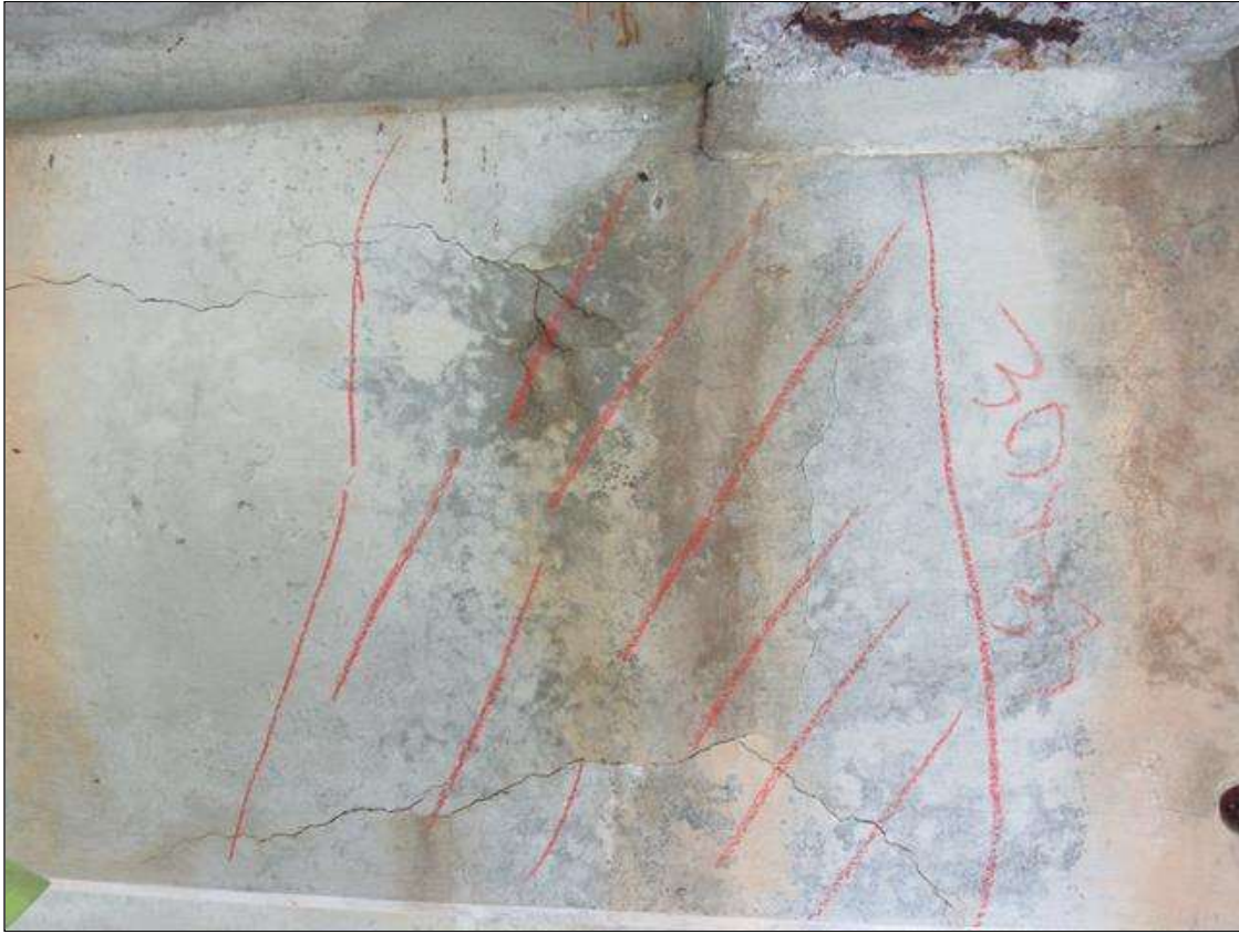
Bent 2 Cap : 0 Feet of Delamination/Spall/Patched Area: Delaminated. Spall 1 inch or less deep or 6 inches or less in diameter. Patched area that is sound BENT 2 EAST FACE OF CAP HAS A CRACKED DELAMINATED AREA AT GIRDER 2 30" X 33".
