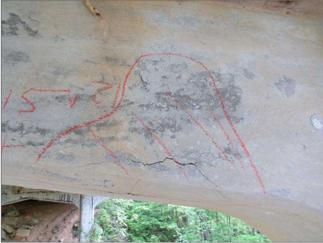
BENT 3 EAST FACE OF HAUNCH AREA LEFT SIDE OF PILE 2 CRACKED AND DELAMINATED 15" UP FACE 21" LONG AND 4" UNDER BOTTOM.
