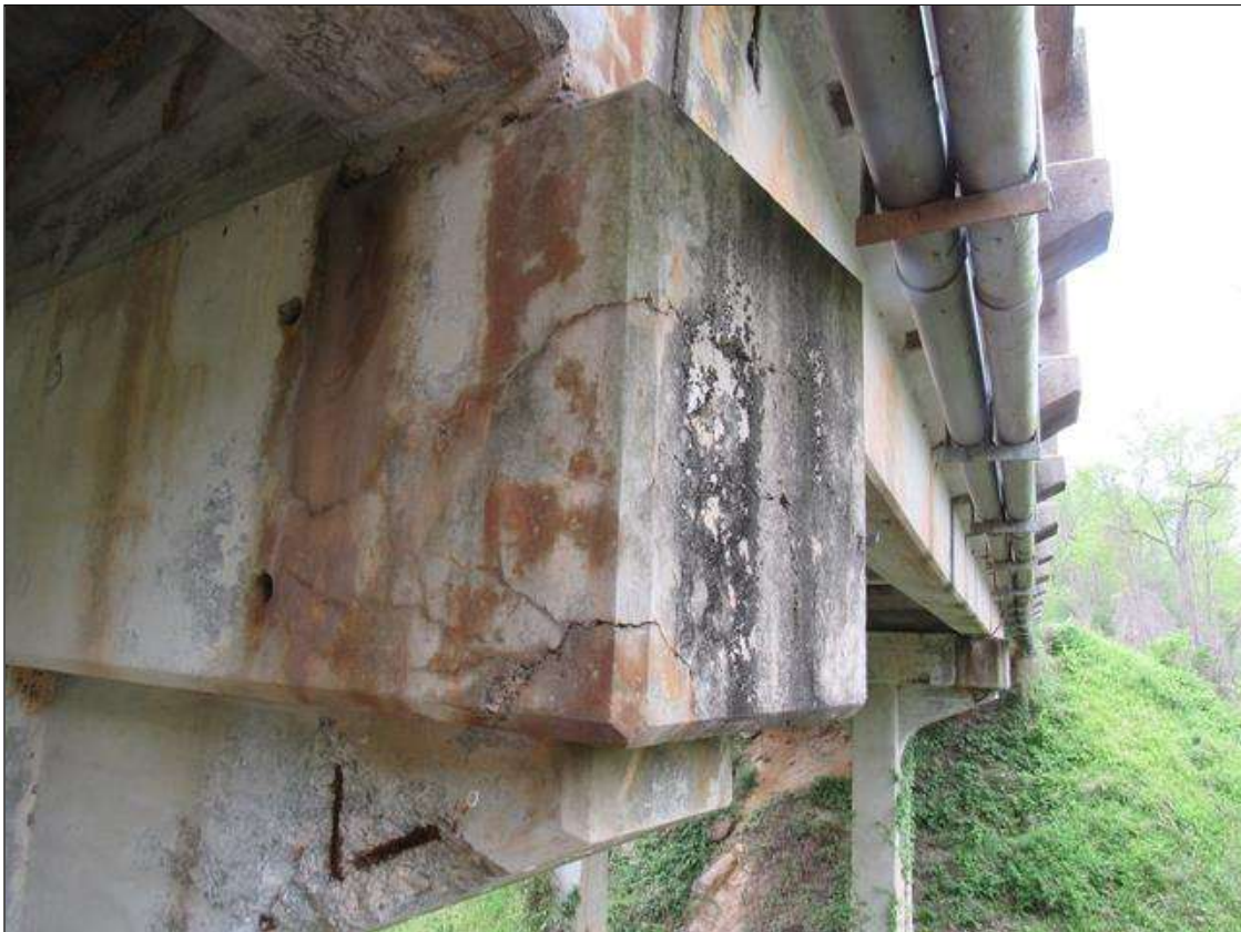
Bent 2 Cap : 0 Feet of Cracking (RC and Other); Width 0.012-0.05 in. or spacing of 1.0-3.0 ft. BENT 2 LEFT END OF CAP MAP CRACKING AND ALONG THE BOTTOM EAST FACE UNDER GIRDER 1.
