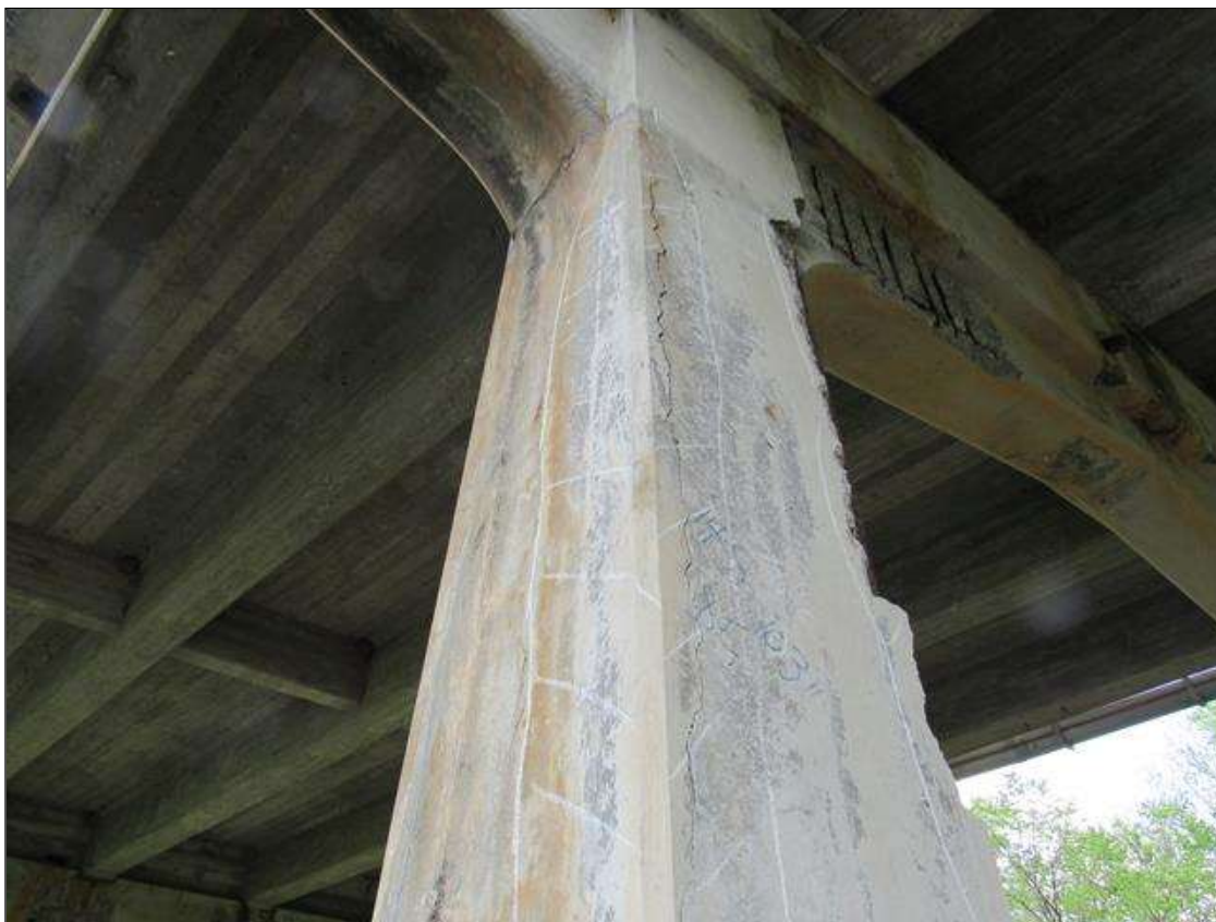
Bent 2 Pile 2: 0 Each of Delamination/Spall/Patched Area: Delaminated. Spall 1 in. or less deep or 6 in. or less in diameter. Patched area that is sound. BENT 2 PILE 2 CRACKED AND DELAMINATED AREA ON SE CORNER OF PILE STARTS 28" BELOW CAP EXTENDS DOWN 103" 14" ON SOUTH FACE AND 8" ON THE EAST.
