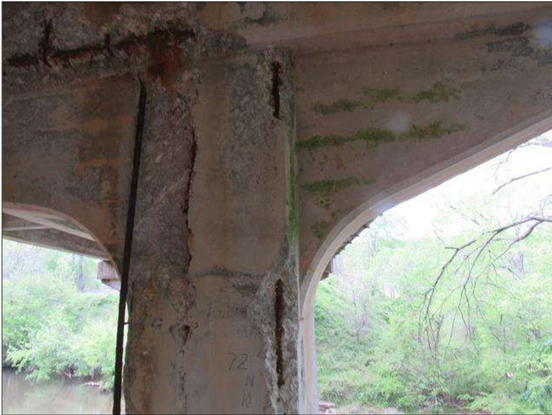
BENT 4 PILE 1 CRACKED SPALL AREA NE CORNER CAP DOWN 72" & 10" ON NORTH FACE & 12" ON EAST WITH REBAR EXPOSED.
