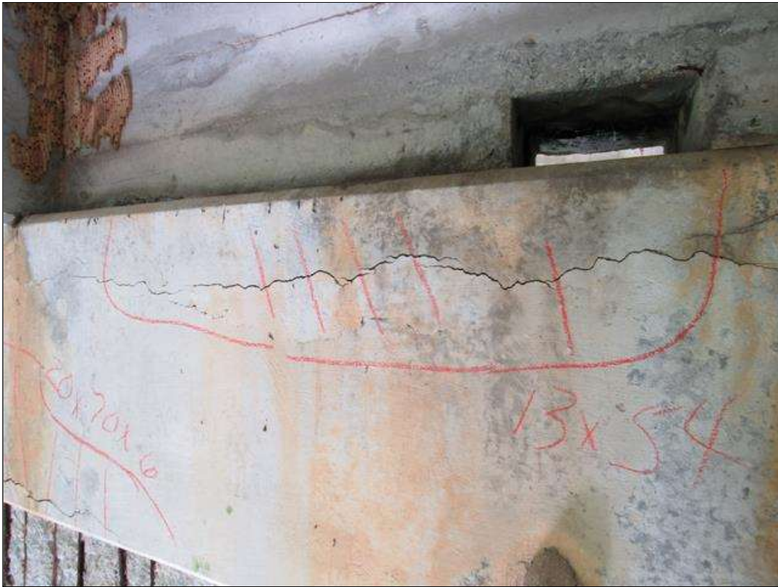
Bent 2 Cap : 0 Feet of Delamination/Spall/Patched Area: Delaminated. Spall 1 inch or less deep or 6 inches or less in diameter. Patched area that is sound BENT 2 EAST FACE OF CAP CRACKED AND DELAMINATED AREA ALONG TOP OF CAP BETWEEN GIRDERS 3 AND 4. 13" X 54".
