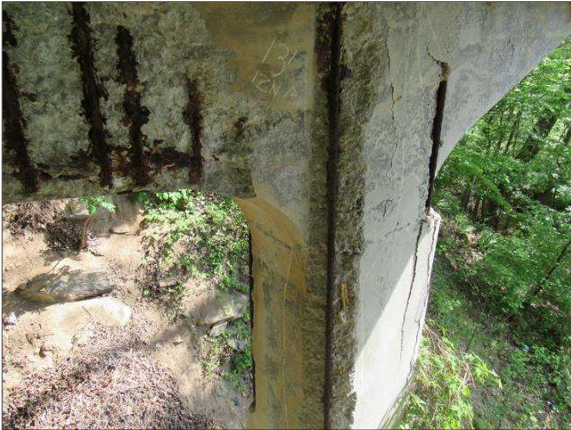
BENT 4 PILE 2 CRACKED SPALL DELAMINATED NW CORNER FM CAP DOWN 13' & 12" ON NORTH FACE 13" ON WEST. REBAR EXPOSED.
