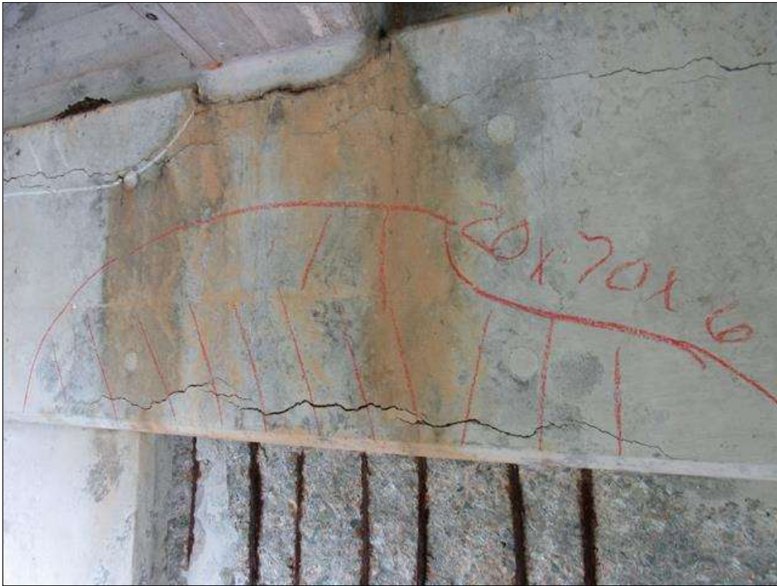
Bent 2 Cap : 0 Feet of Delamination/Spall/Patched Area: Delaminated. Spall 1 inch or less deep or 6 inches or less in diameter. Patched area that is sound BENT 2 EAST FACE OF CAP HAS A CRACKED DELAMINATED AREA ALONG BOTTOM OF CAP UNDER GIRDER 4. 20" UP THE FACE 7" LONG 6" UNDER BOTTOM.
