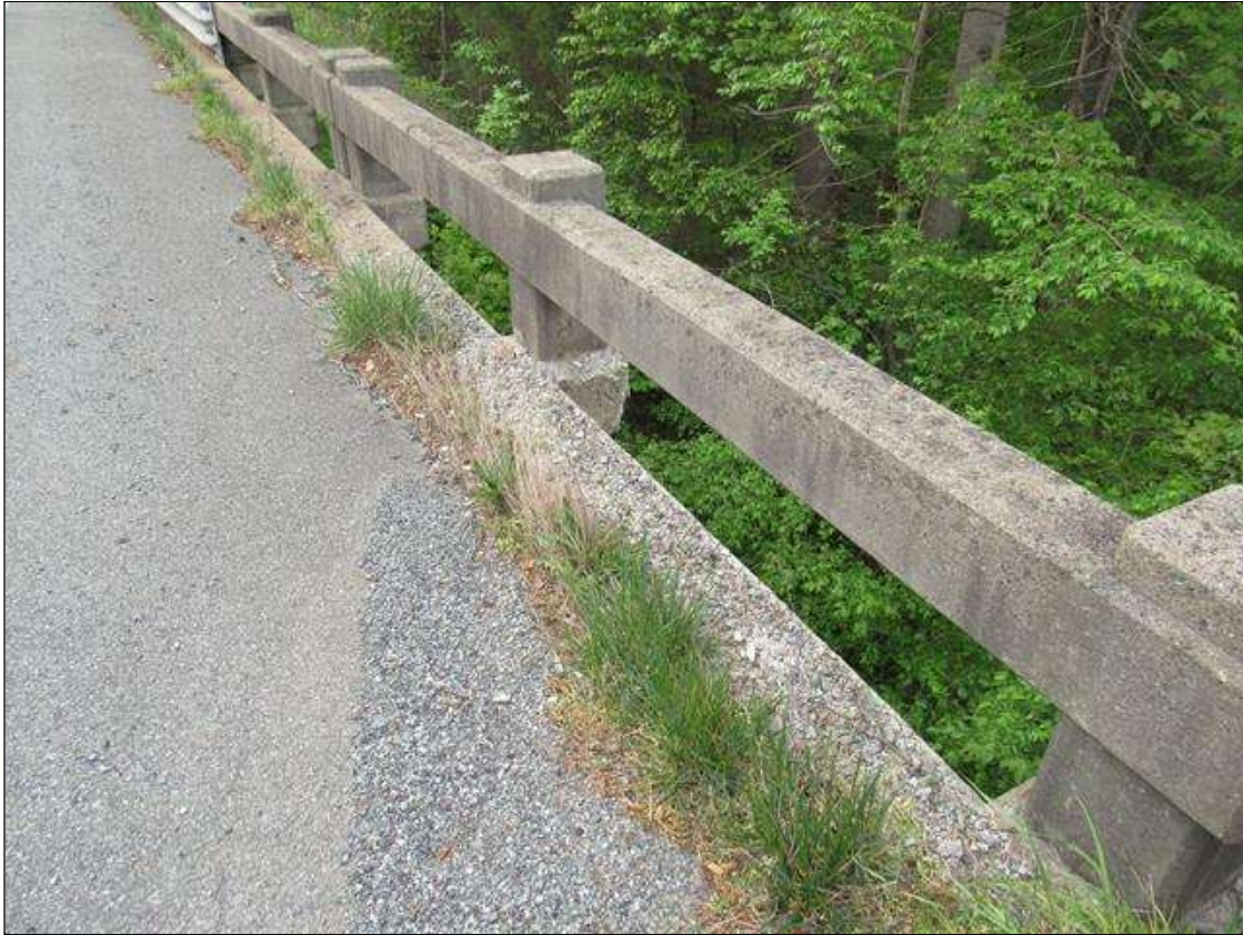
Span 5 Right Bridge Rail: 12 Feet of Delamination/Spall/Patched Area: Spall greater than 1 in. deep or greater than 6 in. diameter. Patched area that is unsound or showing distress. Does not warrant structural review. SPAN 5 RIGHT RAIL POST 2 IS SPALL AND DETERIORATING AND RIGHT CURB CONCRETE IS DETERIORATING FORM JOINT AT BENT 4 OUT TO RAIL POST 3.
