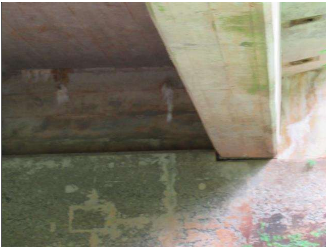
END BENT 2 BACK WALL HAS CRACKS WITH EFFLO IN BAY 4 AND RIGHT SIDE OF G5.
