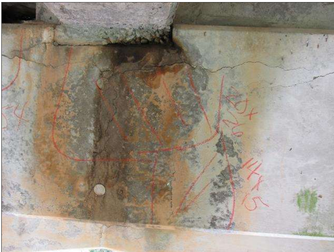
Bent 2 Cap : 0 Feet of Delamination/Spall/Patched Area: Delaminated. Spall 1 inch or less deep or 6 inches or less in diameter. Patched area that is sound BENT 2 EAST FACE OF CAP HAS 2 CRACKED DELAMINATED AREAS UNDER GIRDER 3 14" X 15" AND 20" X 26".
