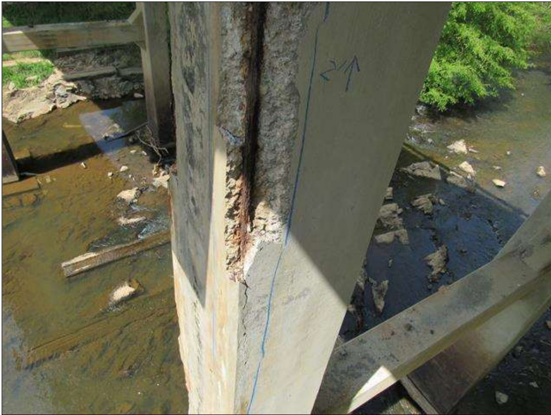
Bent 3 Pile 2: 0 Each of Delamination/Spall/Patched Area: Spall greater than 1 in. deep or greater than 6 in. diameter. Patched area that is unsound or showing distress. Does not warrant structural review. BENT 3 PILE 2 CRACKED SPALL DELAMINATED AREA SE CORNER OF PILE STARTS 24" BELOW CAP EXTENDS DOWN 24' 14" ON SOUTH FACE AND 16" ON EAST LARGE REBAR EXPOSED.
