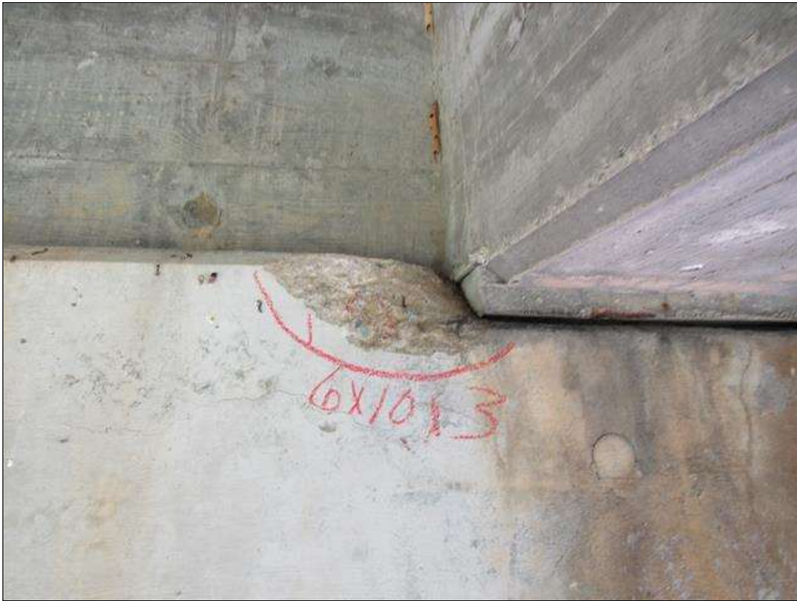
Bent 2 Cap : 1 Feet of Delamination/Spall/Patched Area: Delaminated. Spall 1 inch or less deep or 6 inches or less in diameter. Patched area that is sound BENT 2 CAP WEST FACE HAS A SPALL AREA ALONG LEFT SIDE OF GIRDER 3. 6" X 10" X 3" DEEP.
