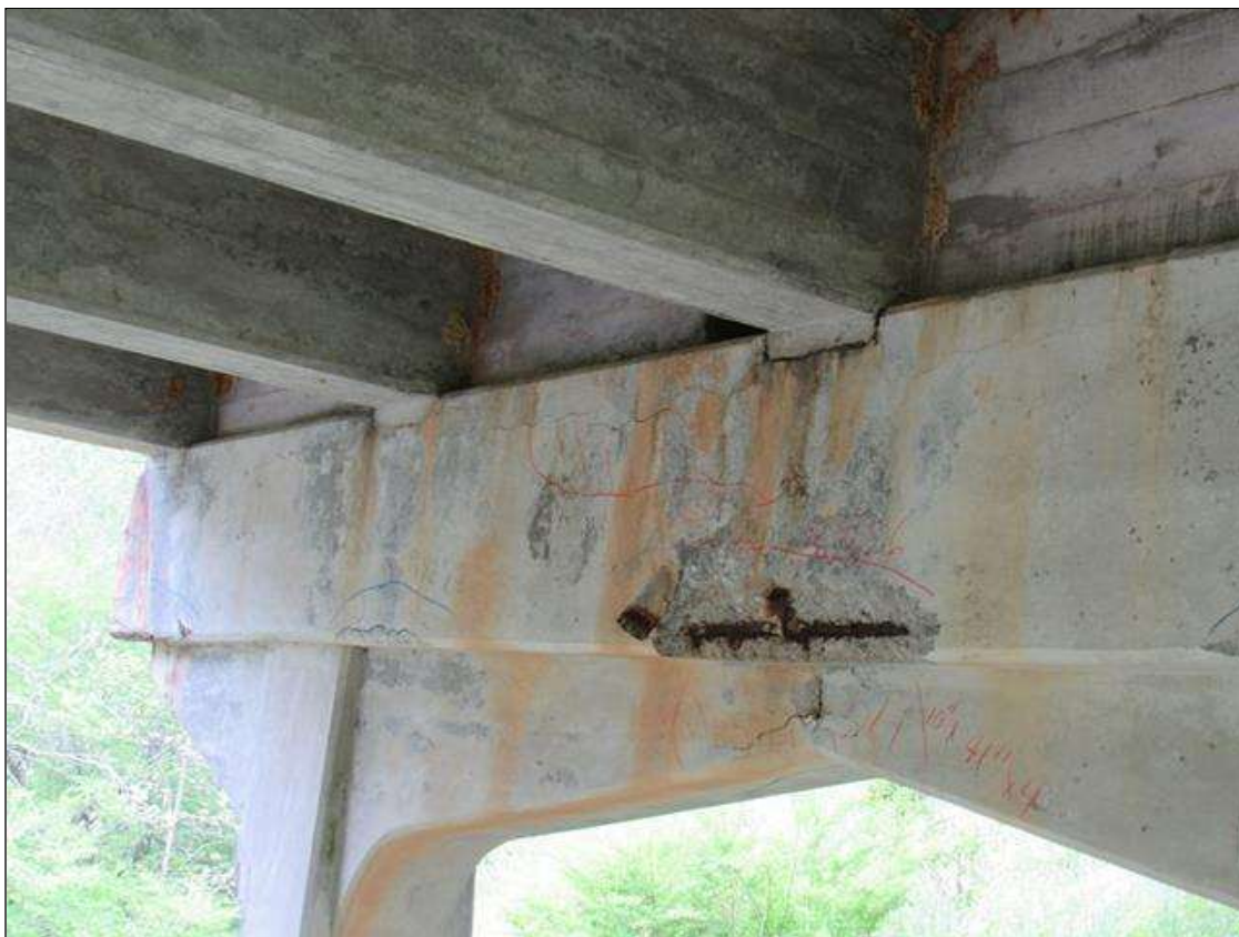
Bent 1 Cap : 0 Feet of Delamination/Spall/Patched Area: Delaminated. Spall 1 inch or less deep or 6 inches or less in diameter. Patched area that is sound BENT 1 EAST FACE OF CAP HAS HORZ CRACKS FROM LEFT TO RIGHT END ALONG THE FACE OF CAP.
