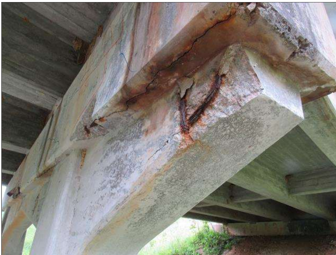
HAUNCH AREA BELOW BOTTOM OF CAP UNDER GIRDER 1 CRCKED SPALL DELAMINATED FM 8" UP FACE 32" LONG AND 12" UNDER BOTTOM.
