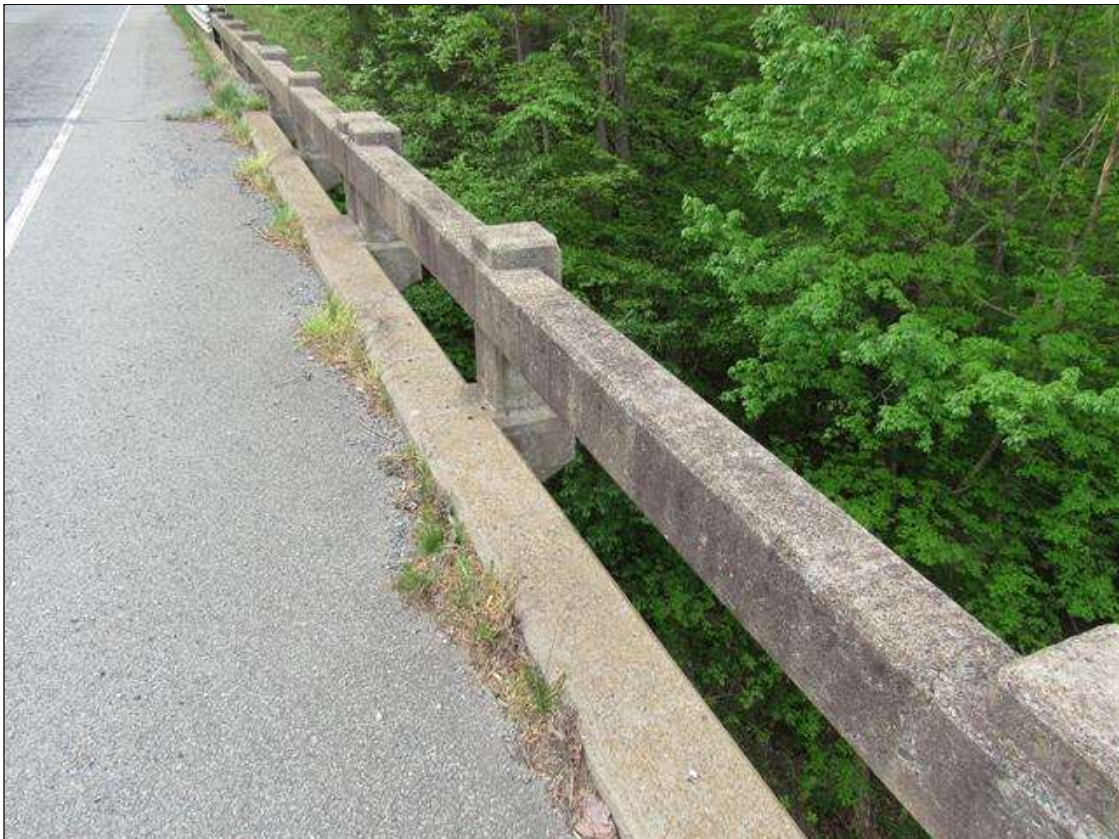
Span 4 Right Bridge Rail: 25 Feet of Cracking (RC and Other): Width 0.012-0.05 in. or spacing of 1.0-3.0 ft. SPAN 4 RIGHT RAIL FINE MAP CRACKING AND SURFACE SCALE ON TOP OF RAIL.
