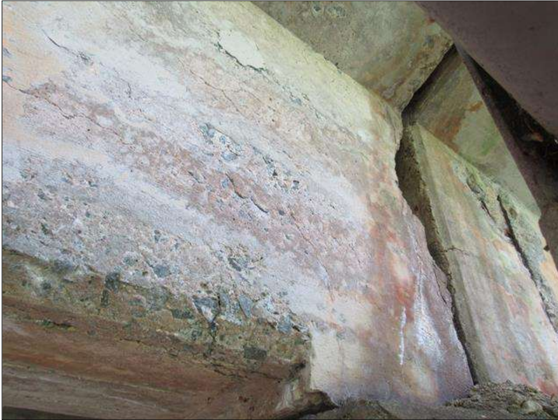
Span 5 Beam 1: 3 Feet of Delamination/Spall/Patched Area: Delaminated. Spall 1 in. or less deep or 6 in. or less in diameter. Patched area that is sound. SPAN 5 LEFT SIDE OF G1 MAP CRACKED AND SPALL AREA ALONG END OF GIRDER OVER BENT 4. SPALL IS 21" DOWN GIRDER 5" WIDE AND 5" DEEP.
