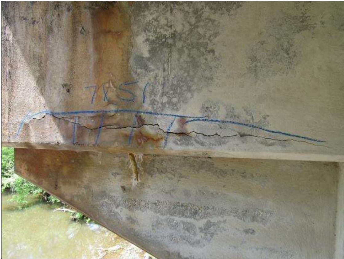
Bent 3 Cap : 0 Feet of Delamination/Spall/Patched Area: Delaminated. Spall 1 inch or less deep or 6 inches or less in diameter. Patched area that is sound BENT 3 EAST FACE OF CAP HAS A CRACKED AND DELAMINATED AREA UNDER GIRDER 5 ALONG THE BOTTOM EDGE. 7" UP FACE AND 51" LONG.
