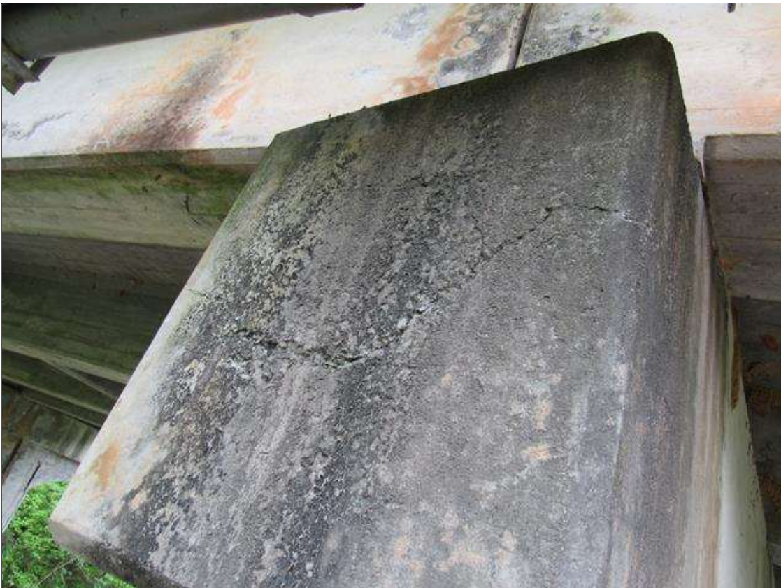
Bent 3 Cap : 0 Feet of Cracking (RC and Other): Width 0.012-0.05 in. or spacing of 1.0-3.0 ft. BENT 3 LEFT END OF CAP IS MAP CRACKED.
