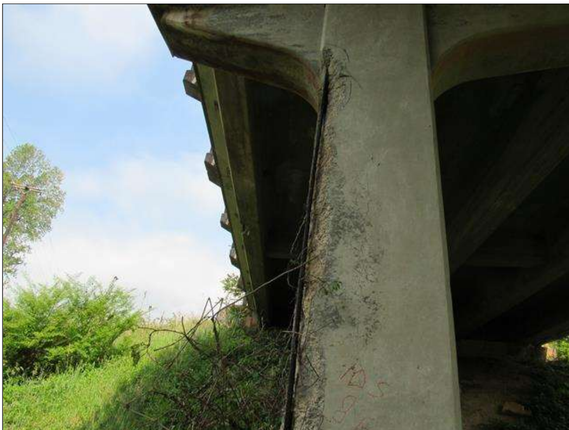
Bent 1 Pile 2: 0 Each of Delamination/Spall/Patched Area: Spall greater than 1 in. deep or greater than 6 in. diameter. Patched area that is unsound or showing distress. Does not warrant structural review. BENT 1 PILE 2 CRACKED SPALL DELAMINATED ON SE CORNER OF PILE 10" ON SOUTH FACE 8" ON EAST 11" DOWN FACE START 32" BELOW THE CAP.
