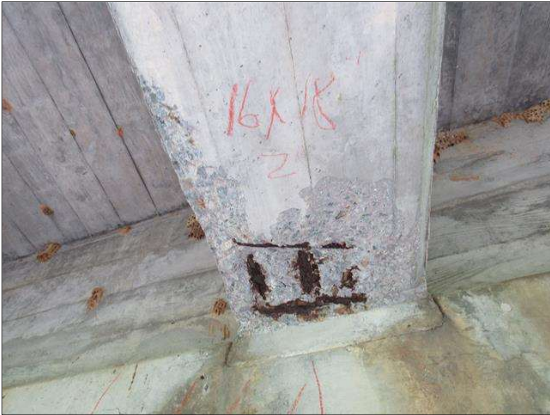
Span 3 Beam 2: 2 Feet of Delamination/Spall/Patched Area: Spall greater than 1 in. deep or greater than 6 in. diameter. Patched area that is unsound or showing distress. Does not warrant structural review. SPAN 3 BEAM 2 AT BENT 2 BOTTOM OF GIRDER HAS A SPALL AREA 16" W FROM CAP OUT 18" AND 2" DEEP REBAR AND STIRRUPS EXPOSED.
