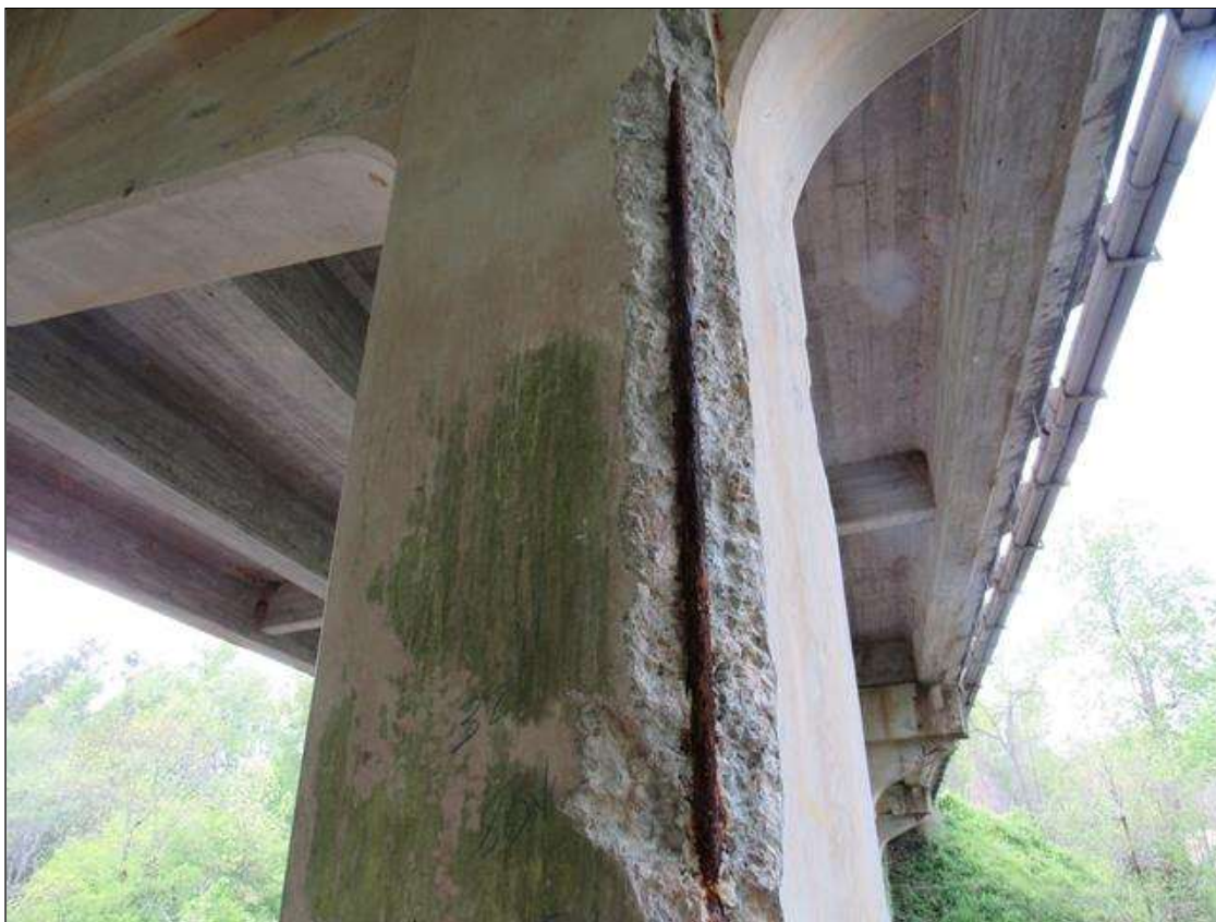
Bent 3 Pile 1: 0 Each of Delamination/Spall/Patched Area: Spall greater than 1 in. deep or greater than 6 in. diameter. Patched area that is unsound or showing distress. Does not warrant structural review. BENT 3 PILE 1 CRACKED SPALL DELAMINATED AREA NE CORNER OF PILE STARTS 32" BELOW CAP EXTENDS DOWN 80" 11" ON EAST AND 6" NORTH.
