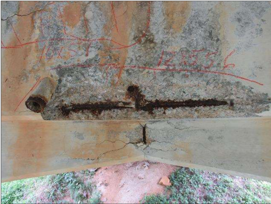
Bent 1 Cap : 0 Feet of Delamination/Spall/Patched Area: Spall greater than 1 inch deep or greater than 6 inches in diameter. Patched area that is unsound or showing distress. Condition does not warrant structural Review BENT 1 EAST OF CAP HAS CRACKED SPALL DELAMINATED AREA ALONG BOTTOM EDGE OF CAP UNDER GIRDER 3. 12" UP FACE 15" LONG 6" UNDER BOTTOM REBAR AND STIRRUPS EXPOSED.
