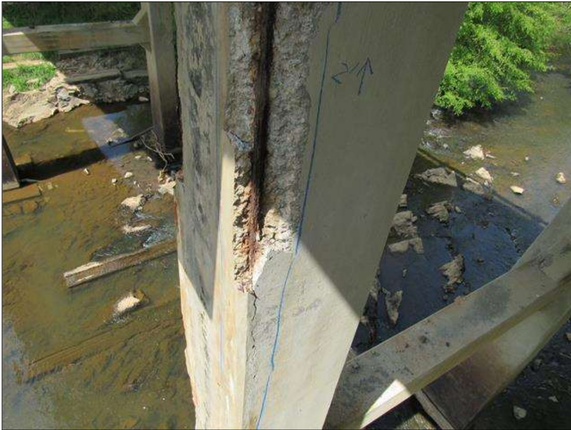
BENT 3 PILE 2 CRACKED SPALL DELAMINATED AREA SE CORNER OF PILE STARTS 24" BELOW CAP EXTENDS DOWN 24' 14" ON SOUTH FACE AND 16" ON EAST LARGE REBAR EXP
