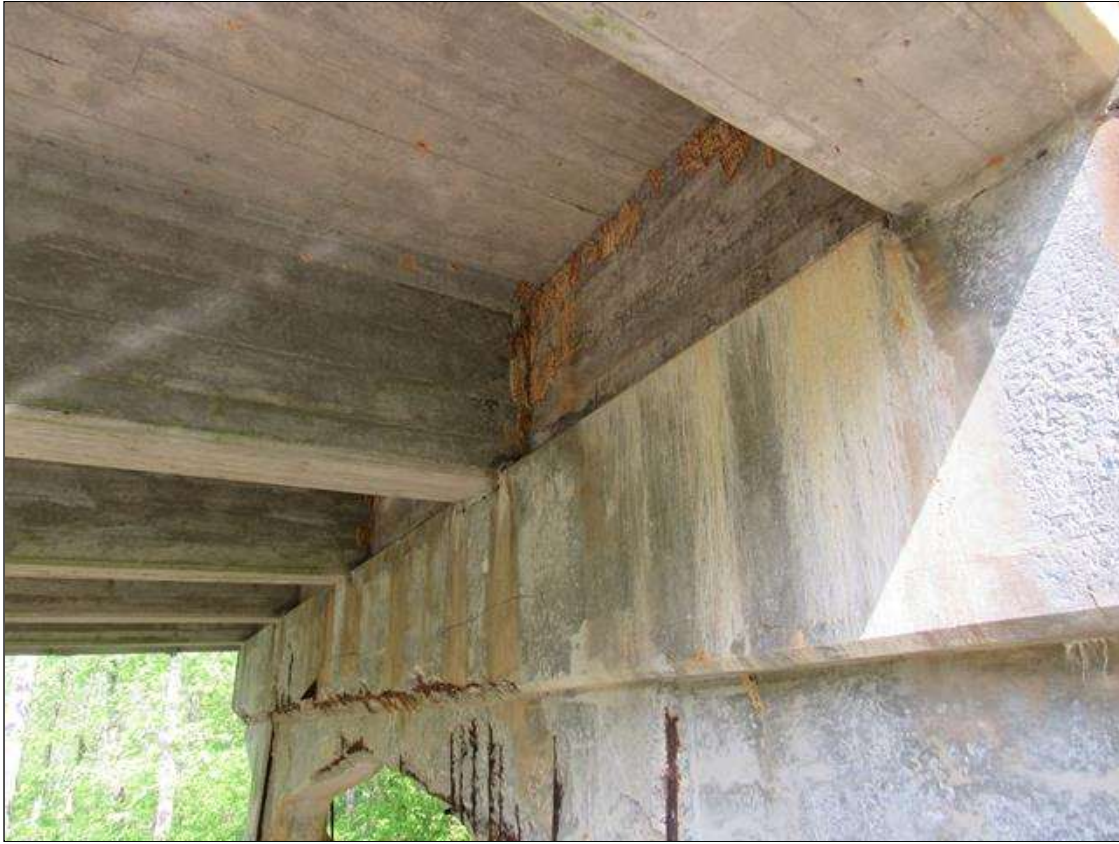
Bent 4 Cap : 7 Feet of Cracking (RC and Other): Width 0.012-0.05 in. or spacing of 1.0-3.0 ft. BENT 4 WEST FACE OF CAP HORZ CRACK ALONG TOP EDGE FM G1 TO G4 WITH EFFLO ON FACE OF CAP LEFT SIDE OF G5.
