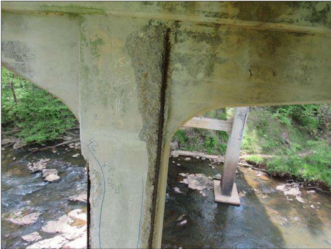
BENT 2 PILE 1 HAS A CRACKED SPALL DELAM AREA ON SW CORNER FM BOTTOM OF CAP DOWN 16' 5" FROM 8 TO 15 ON WEST FACE AND 10" ON SOUTH. LARGE REBAR EXPOSED
