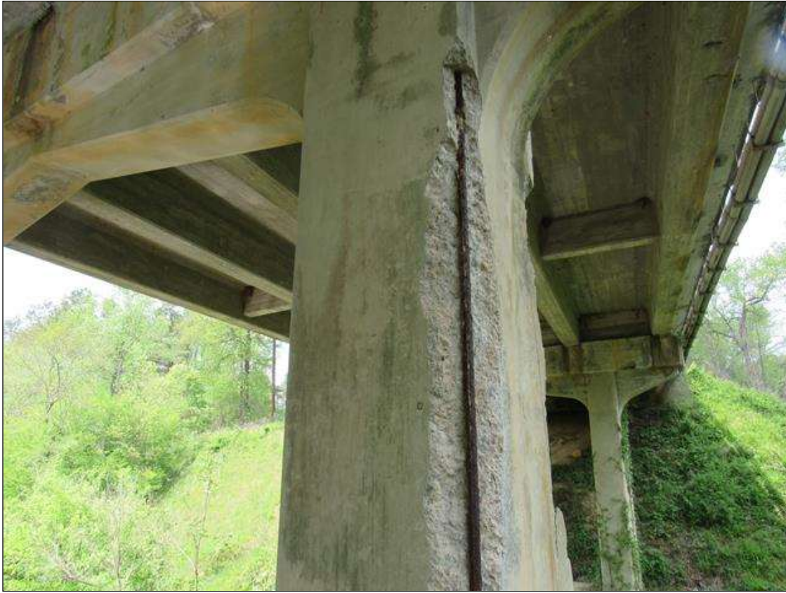
Bent 1 Pile 1: 0 Each of Delamination/Spall/Patched Area: Spall greater than 1 in. deep or greater than 6 in. diameter. Patched area that is unsound or showing distress. Does not warrant structural review. BENT 2 PILE 1 NE CORNER CRACKED SPALL DELAMINATED STARTS 3' BELOW CAP EXTENDS DOWN 7' 9" ON EACH FACE. LARGE REBAR EXPOSED.
