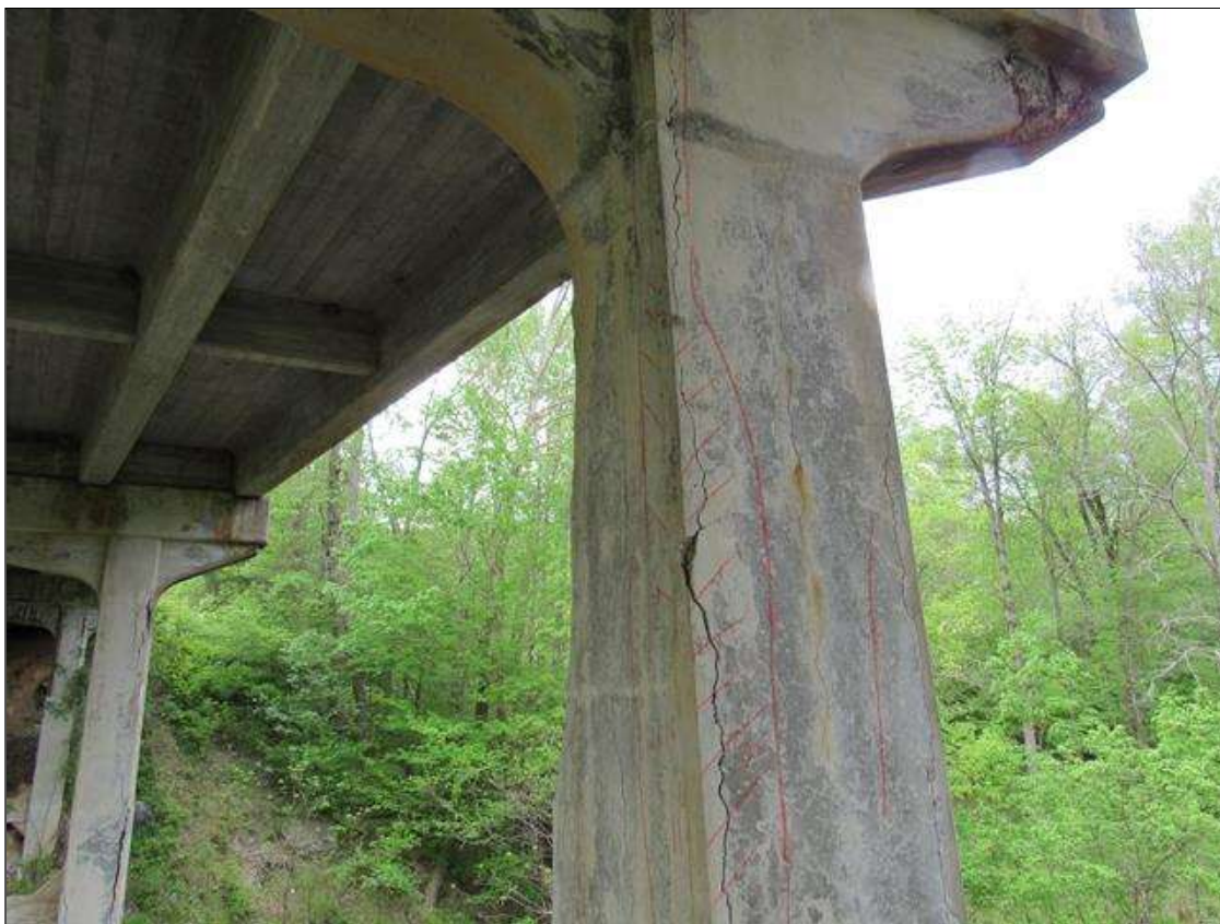
Bent 2 Pile 2: 1 Each of Delamination/Spall/Patched Area: Delaminated. Spall 1 in. or less deep or 6 in. or less in diameter. Patched area that is sound. BENT 2 PILE 2 CRACKED DELAMINATED AREA ON NW FACE OF PILE FM TOP DOWN 11' AND 11" ON NORTH AND 9" ON WEST.
