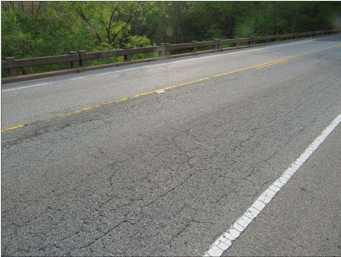
Span 2 Wearing Surface: 1615 Square Feet of Crack (Wearing Surface): Width 0.012-0.05 in. or spacing of 1.0-3.0 ft. SPAN 2 WEARING SURFACE HEAVILY MAP CRACKED BOTH LEFT AND RIGHT LANES.
