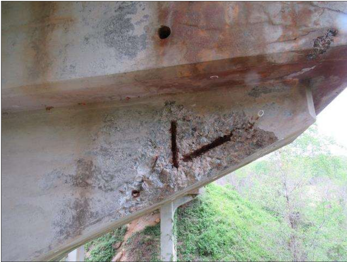
HAUNCH AREA ON EAST FACE OF BENT 2 UNDER GIRDER 1 IS SPALL WITH REBAR EXPOSED. 13" X 28" X 2" DEEP.
