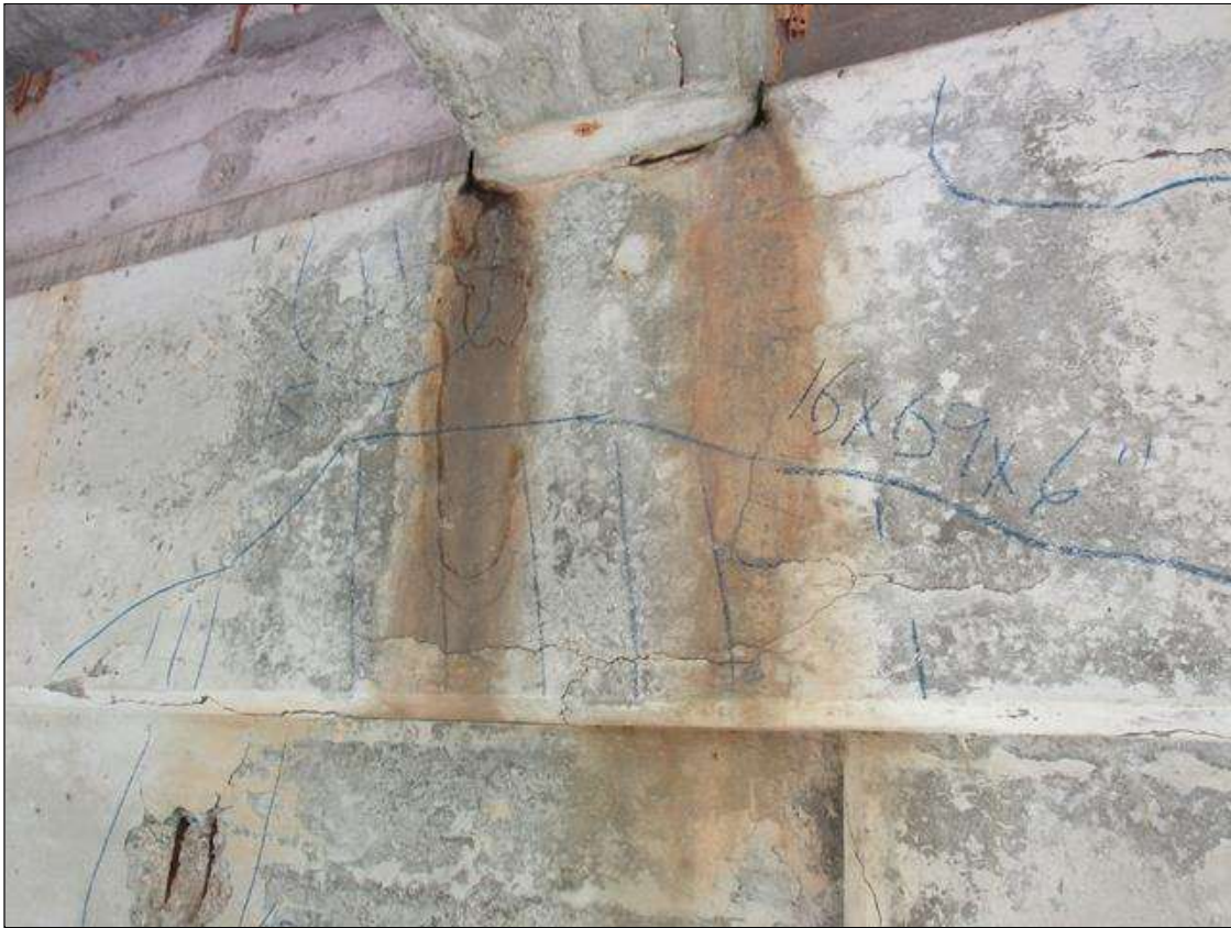
Bent 1 Cap : 0 Feet of Delamination/Spall/Patched Area: Delaminated. Spall 1 inch or less deep or 6 inches or less in diameter. Patched area that is sound BENT 1 EAST FACE OF CAP HAS 2 SPALL AREAS UNDER GIRDER 2 15' X 16" AND FM BOTTOM UP 16" 69" LONG AND 6" UNDER BOTTOM.
