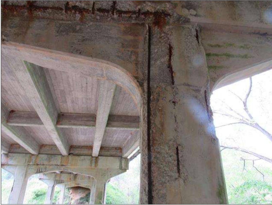
Bent 4 Pile 1: 0 Each of Delamination/Spall/Patched Area: Spall greater than 1 in. deep or greater than 6 in. diameter. Patched area that is unsound or showing distress. Does not warrant structural review. BENT 4 PILE 1 CRACKED SPALL DELAMINATED AREA ON SE CORNER OF PILE FM CAP DOWN 9' 4" AND 10" ON SOUTH 15" ON EAST REBAR EXPOSED.
