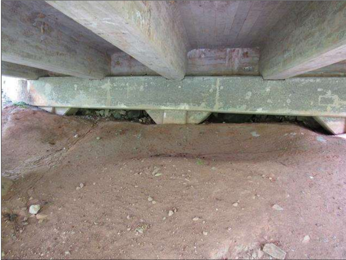
END BENT 2 ERROSION AREA UNDER BOTTOM OF CAP FROM PILE 1 TO PILE 3 12" TO 15" UNDER BOTTOM AND 36" BACK.
