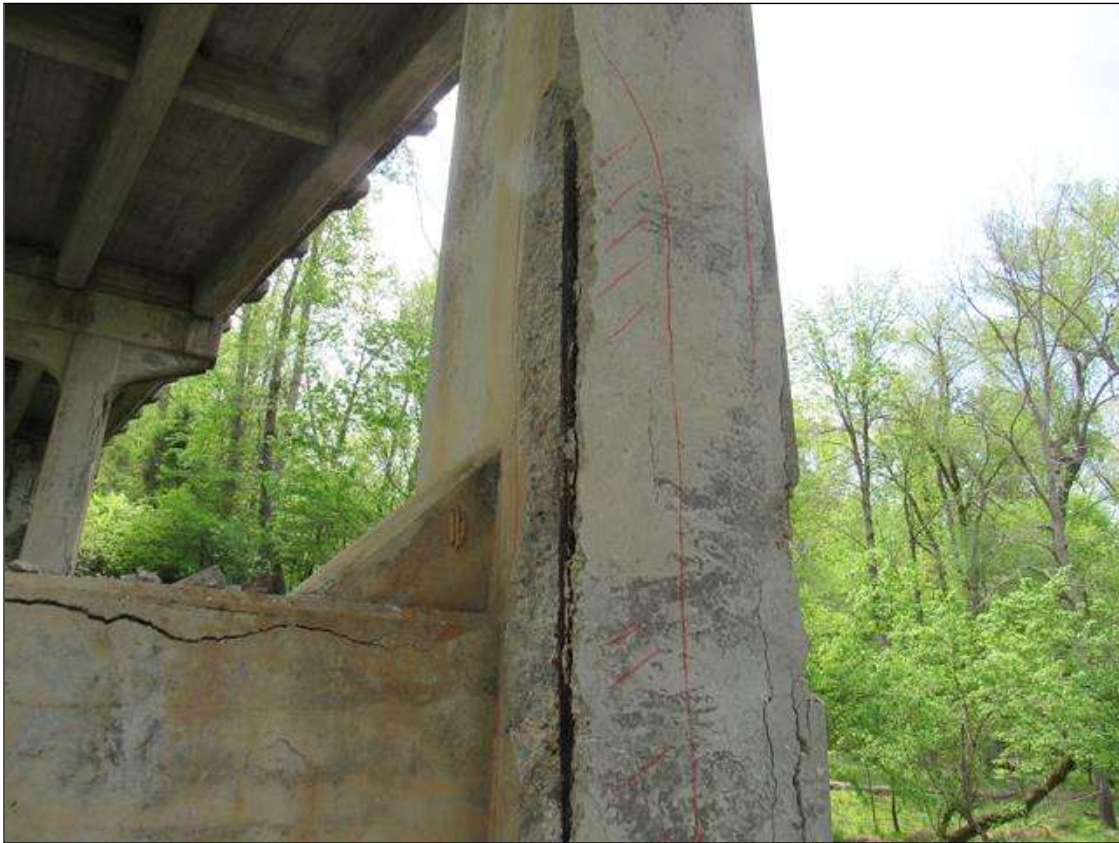
DELAMINATED AREA NW CORNER 10" ON NORTH 12 ON WEST, START 14' ABOVE FOOTING EXTENDS UP 9' HIGH WITH LARGE REBAR EXPOSED.
