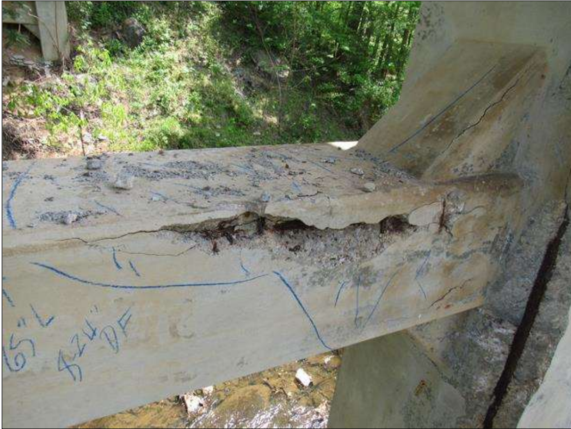
BENT 3 HORZ STRUT AREA LEFT SIDE OF PILE 2 IS CRACKED SPALL DELAMINATED 24" ON TOP 65" LONG AND FROM 8" TO 24" DOWN FACE REBAR AND STIRRUPS EXPOSED.
