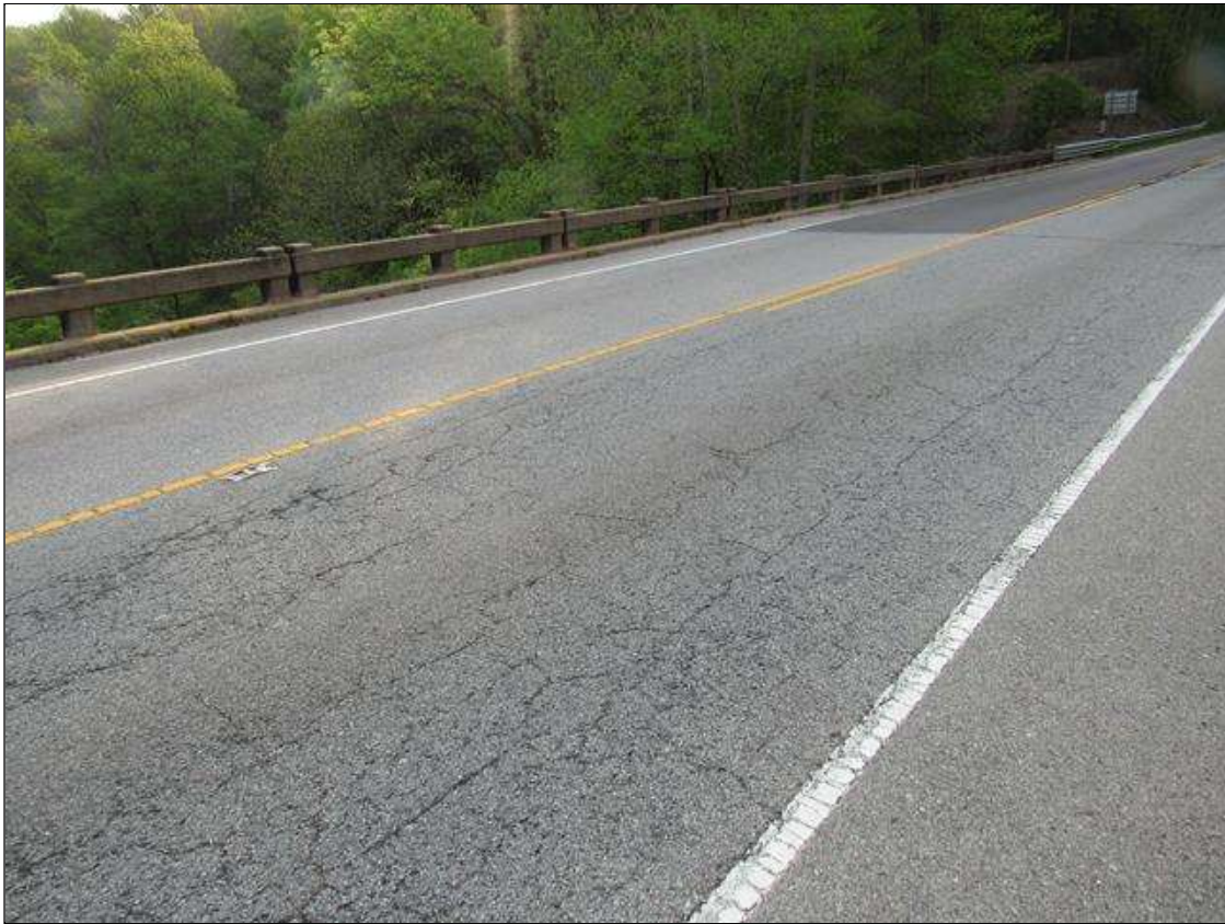
Span 3 Wearing Surface: 1615 Square Feet of Crack (Wearing Surface): Width 0.012-0.05 in. or spacing of 1.0-3.0 ft. SPAN 3 WEARING SURFACE IS HEAVILY MAP CRACKED IN BOTH LEFT AND RIGHT LANES.
