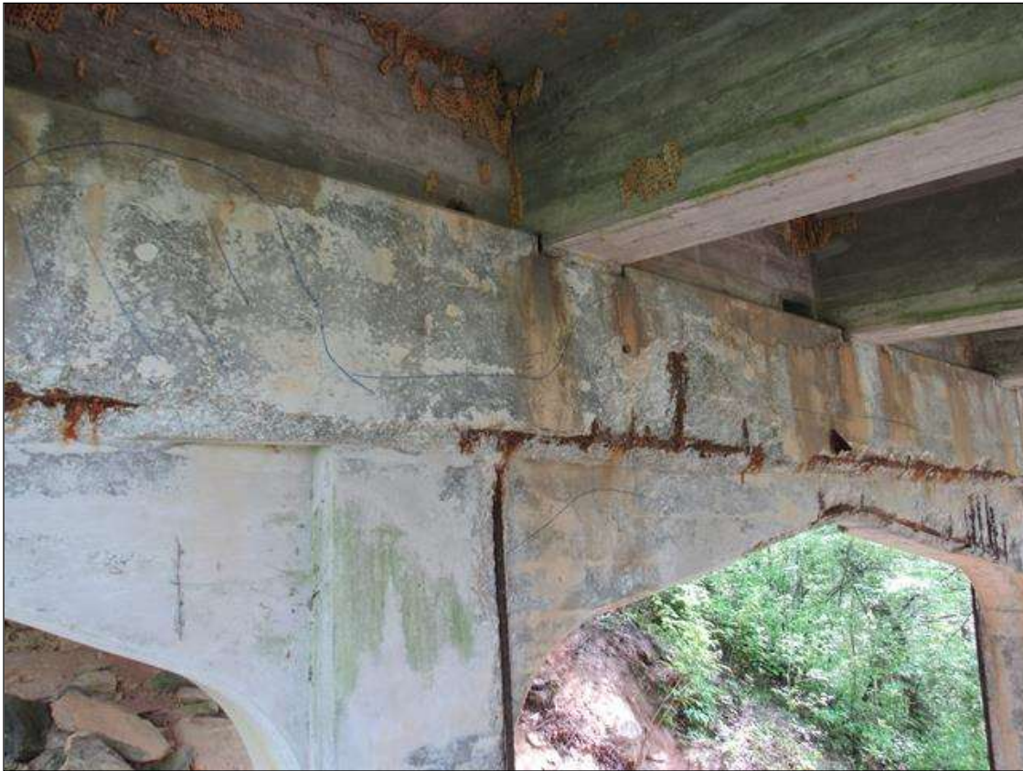
BENT 4 WEST FACE OF CAP FM LT END OVER TO PILE 2 CRACKED SPALL DELAMINATED 27' LONG FM 12' TO 30" FM BOTTOM OF CAP UP WITH REBAR AND STIRRUPS EXPOSED.
