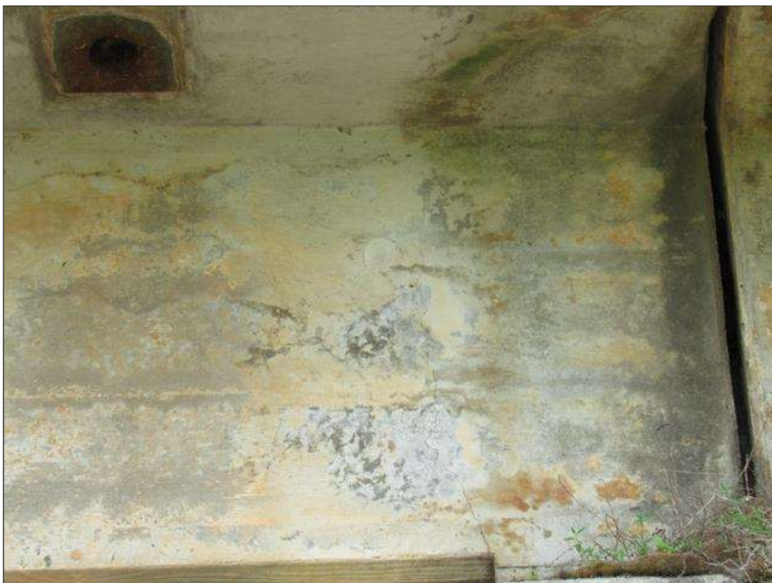
Span 3 Beam 5: 3 Feet of Cracking (RC and Other): Width 0.012-0.05 in. or spacing of 1.0-3.0 ft. SPAN 3 RIGHT SIDE OF GIRDER 5 MAP CRACKING OVER BENT 3 CAP.
