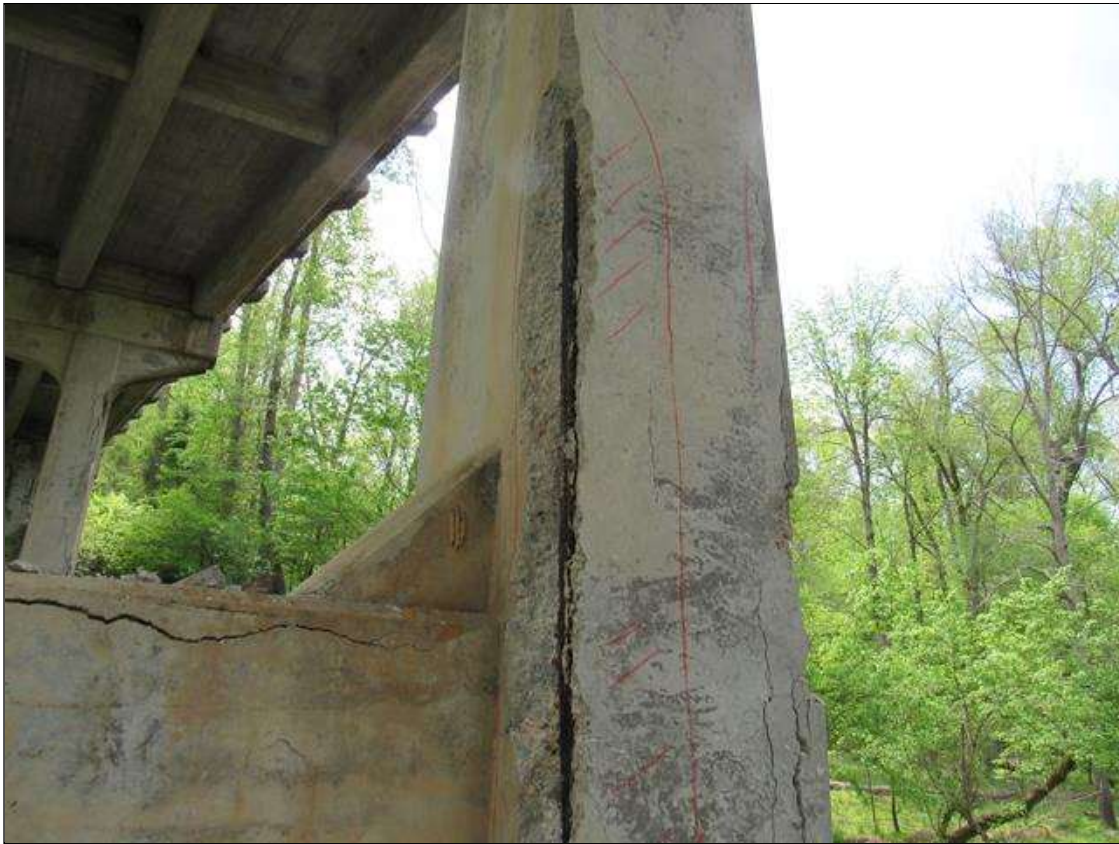
Bent 2 Pile 2: 0 Each of Delamination/Spall/Patched Area: Spall greater than 1 in. deep or greater than 6 in. diameter. Patched area that is unsound or showing distress. Does not warrant structural review. BENT 2 PILE 2 HAS A CRACKED SPALL DELAMINATED AREA NW CORNER 10" ON NORTH 12 ON WEST, START 14' ABOVE FOOTING EXTENDS UP 9' HIGH WITH LARGE REBAR EXPOSED.
