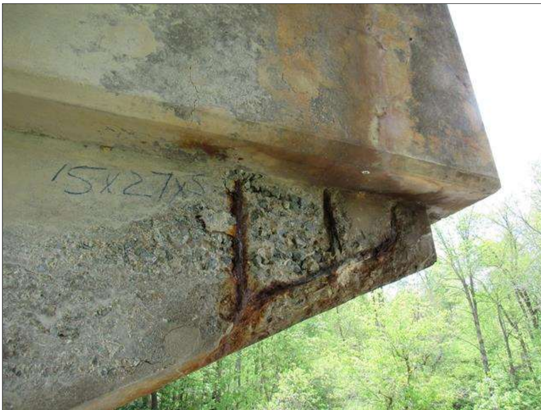
BENT 2 WEST FACE OF HAUNCH AREA UNDER GIRDER 5 CRACKED SPALL AND DELAMINATED. 15" DOWN THE FACE 27" LONG AND 5" UNDER BOTTOM WITH REBAR AND STIRRUPS EXPOSED.
