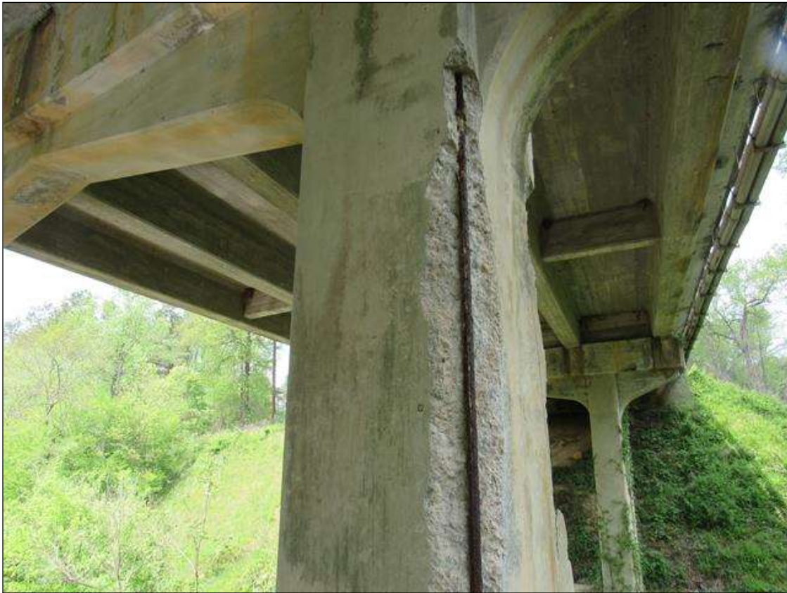
BENT 2 PILE 1 NE CORNER CRACKED SPALL DELAMINATED STARTS 3' BELOW CAP EXTENDS DOWN 7' 9" ON EACH FACE. LARGE REBAR EXPOSED.
