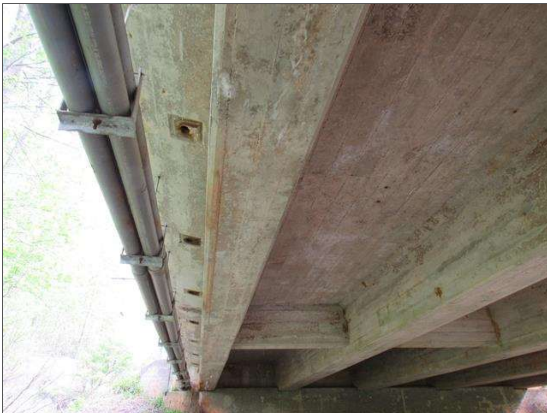
Span 5 Beam 1: 30 Feet of Cracking (RC and Other): Width 0.012-0.05 in. or spacing of 1.0-3.0 ft. SPAN 5 BOTTOM OF G1 FROM BENT 4 TO END BENT 2 SCATTERED LONGITUDINAL CRACKS WITH EFFLO STAINS.
