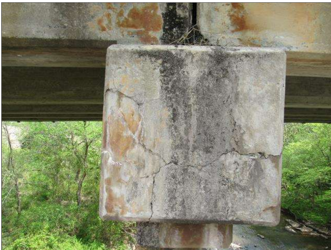
Bent 2 Cap : 0 Feet of Cracking (RC and Other): Width greater than 0.05 in. or spacing of less than 1 ft. BENT 2 CAP RIGHT END OF CAP HEAVILY MAP CRACKED.
