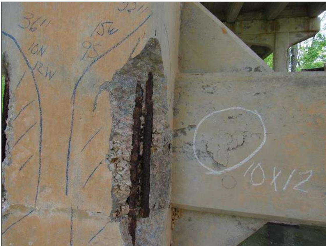
BENT 2 PILE 1 CRCKED SPALL DELAM AREA ON SW CORNER OF PILE STARTS 14' ABOVE FOTING EXTEND UP 52" 15" ON WEST FACE AND 9" ON SOUTH WITH 2 LRGE REBAR EX
