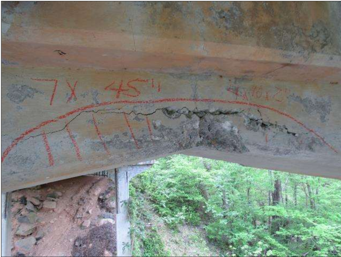
BENT 3 EAST FACE OF THE HAUNCH UNDER GIRDER 3 CRACKED SPALL AND DELAMINATED. 7" X 45" AND SPALL AREA IS 7" X 10" X 2" DEEP.
