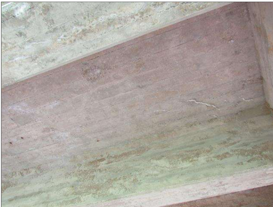
Span 5 Deck: 350 Square Feet of Cracking (RC and Other): Width 0.012-0.05 in. or spacing of 1.0-3.0 ft. SPAN 5 BOTTOM OF DECK HAS SCATTERED MAP CRACKING WITH EFFLO THROUGH OUT BAY 1.
