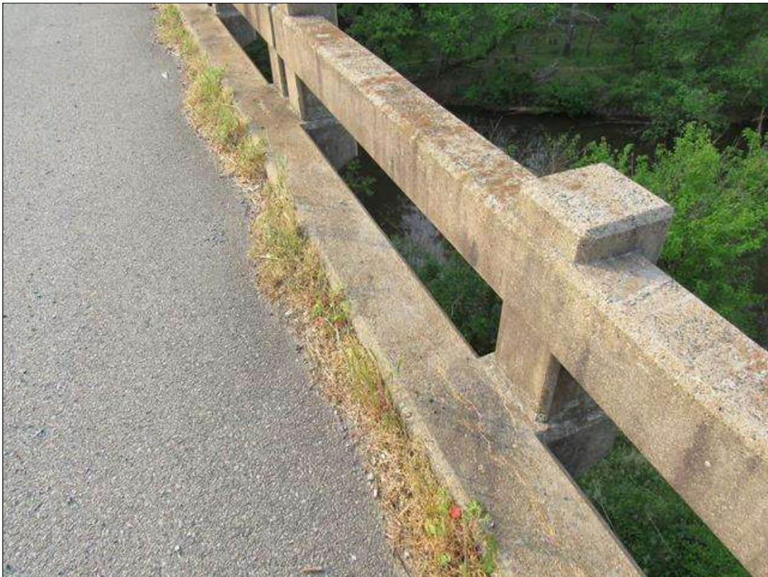
Span 1 Right Bridge Rail: 15 Feet of Cracking (RC and Other): Width 0.012-0.05 in. or spacing of 1.0-3.0 ft. SPAN 1 RIGHT RAIL AND CURB CRACKING WITH SURFACE SCALE.
