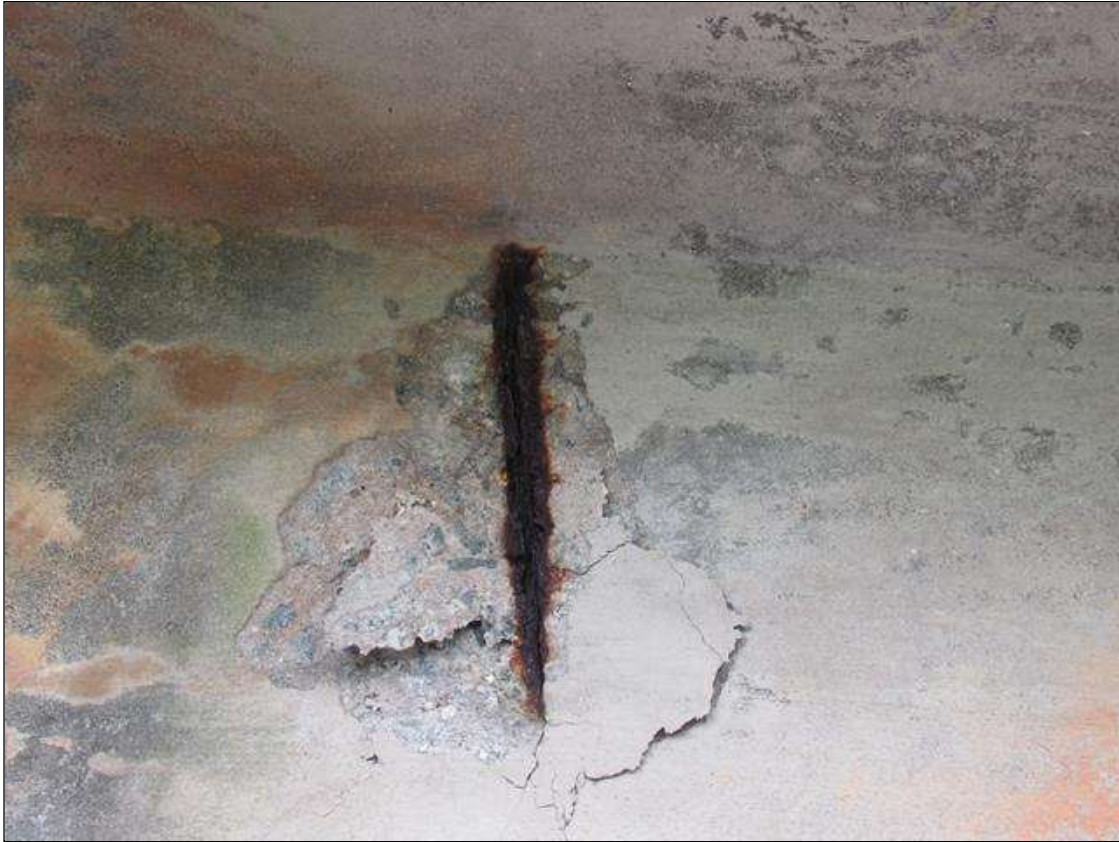
Span 2 Beam 1: 1 Feet of Delamination/Spall/Patched Area: Delaminated. Spall 1 in. or less deep or 6 in. or less in diameter. Patched area that is sound. SPAN 2 GIRDER 1 LEFT SIDE OVER BENT 2 HAS A 9" X 10" SURFACE SPALL AREA 3/4" DEEP WITH REBAR EXPOSED.
