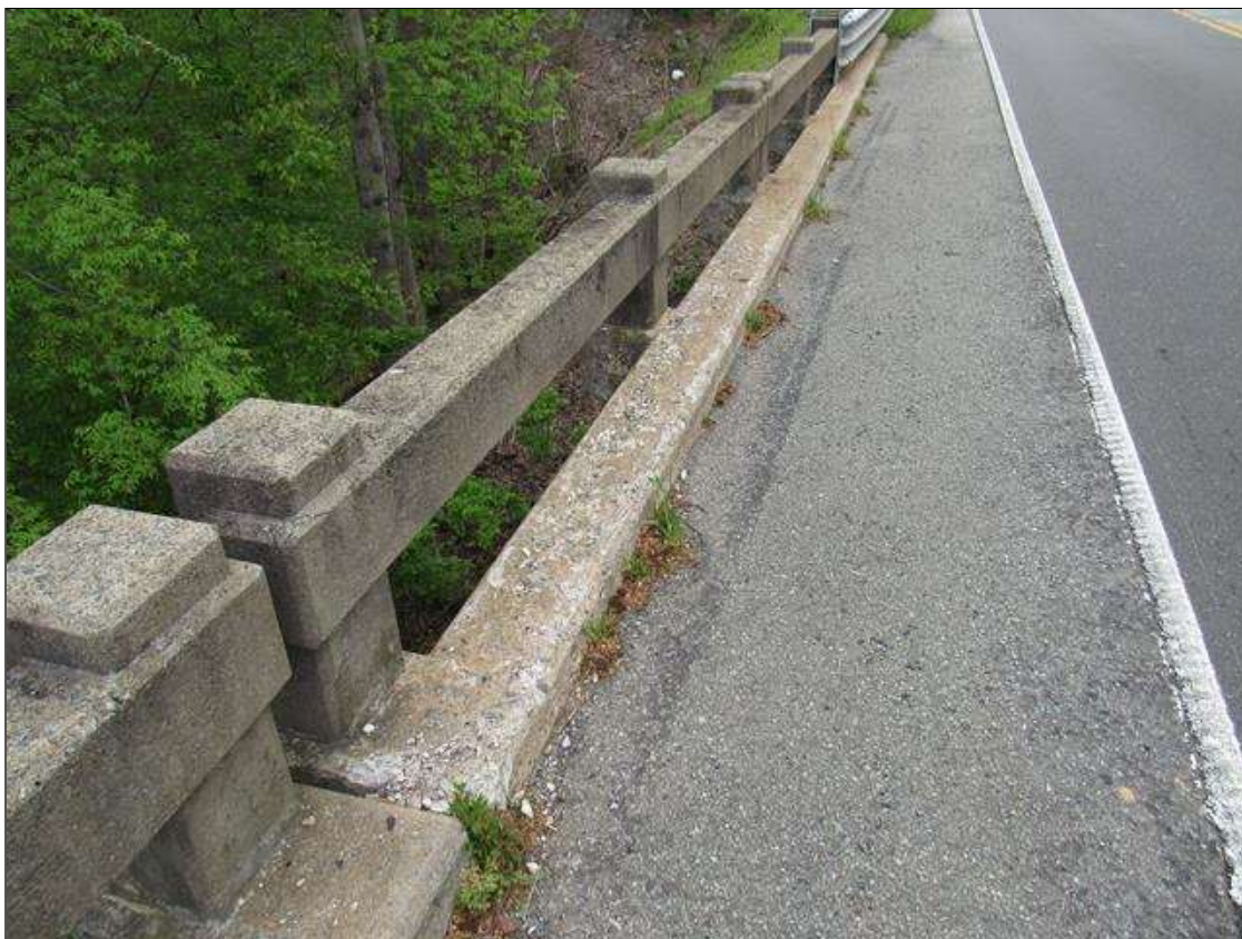
Span 5 Left Bridge Rail: 48 Feet of Cracking (RC and Other): Width greater than 0.05 in. or spacing of less than 1 ft. SPAN 5 LEFT RAIL MAP CRACKING AND SURFACE DETERIORATION FROM BENT 4 TO END OF BRIDGE.
