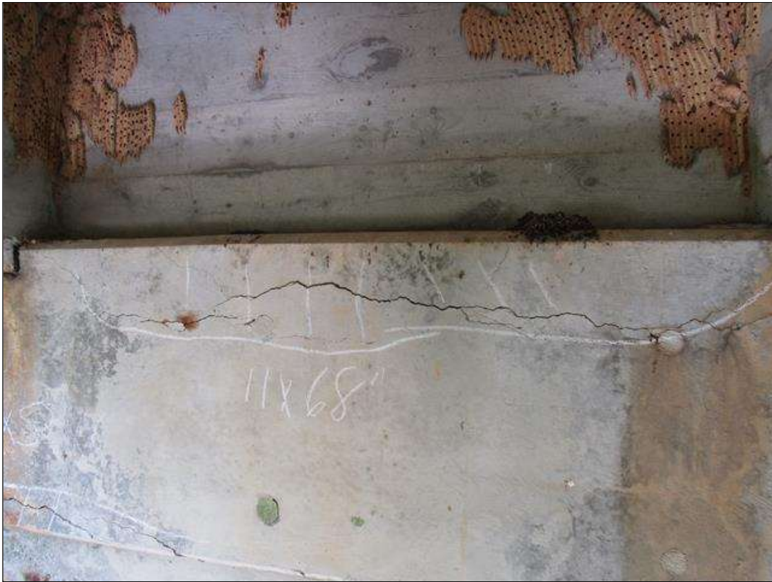
Bent 2 Cap : 6 Feet of Delamination/Spall/Patched Area: Delaminated. Spall 1 inch or less deep or 6 inches or less in diameter. Patched area that is sound BENT 2 EAST FACE OF CAP HAS A CRACKED DELAMINATED AREA BETWEEN G1 AND G5 11" DOWN FACE AND 60" LONG.
