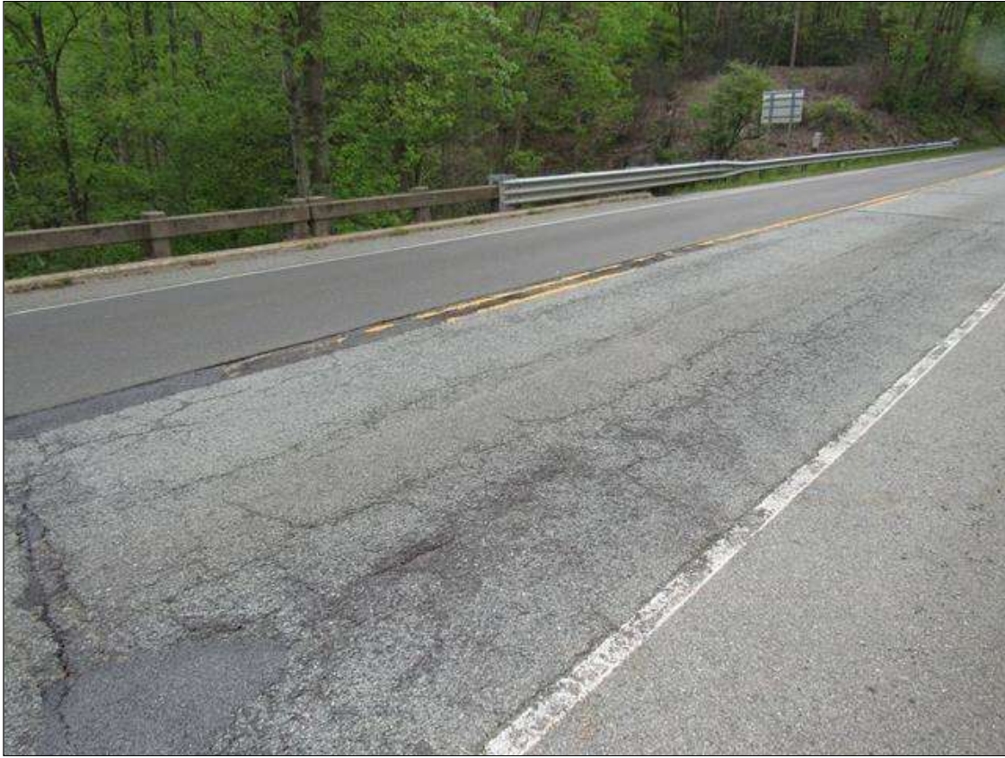
Span 5 Wearing Surface: 1615 Square Feet of Crack (Wearing Surface): Width 0.012-0.05 in. or spacing of 1.0-3.0 ft. SPAN 5 WEARING SURFACE HEAVILY MAP CRACKED ON TOP.
