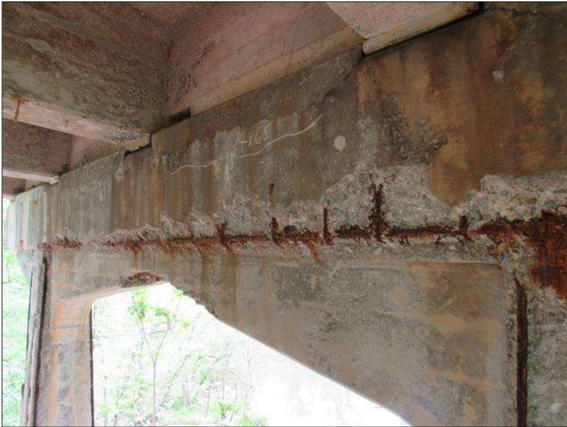
BENT 4 CAP EAST FACE OF CAP CRACKED SPALL DELAM FM LEFT SIDE OF G2 TO RIGHT OF G4. 17" UP FACE 21' LONG 6" UNDER BOTTOM REBAR AND STIRRUPS EXPOSED.
