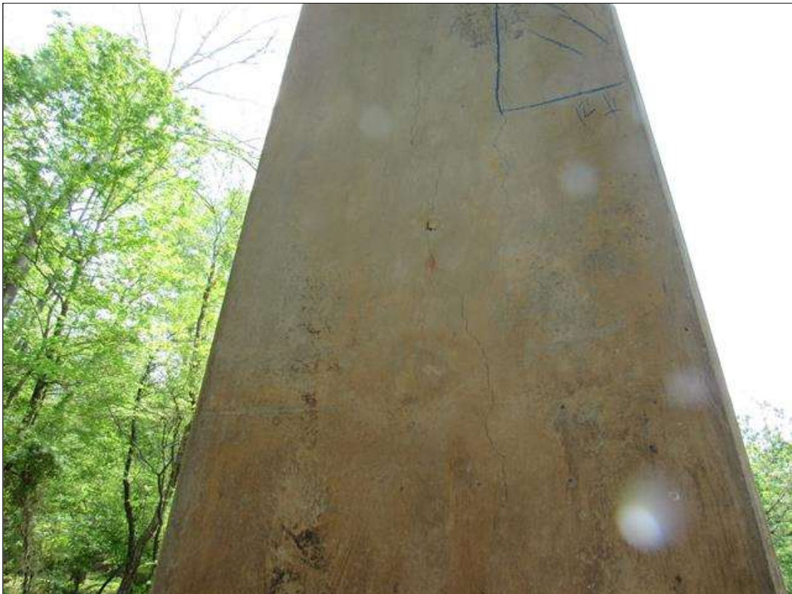
Bent 3 Pile 2: 1 Each of Cracking (RC and Other): Width 0.012-0.05 in. or spacing or 1.0-3.0 ft. BENT 3 PILE 2 HAS SCATTERED VERTICAL CRACKS IN FACE OF PILE.
