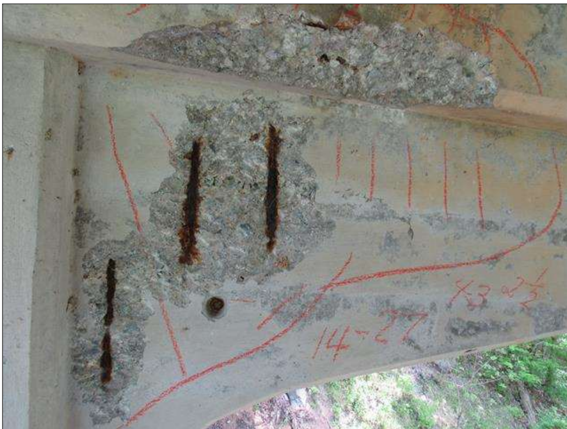
BENT 3 WEST FACE OF HAUNCH RIGHT SIDE OF PILE 1 CRACKED SPALL DELAMINATED. 14" TO 27" DOWN FACE 43" LONG 2 1/2" DEEP REBAR EXPOSED.
