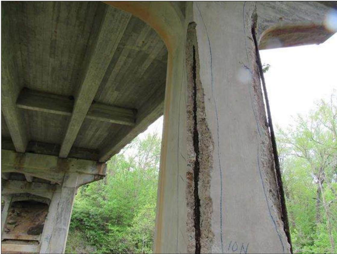
BENT 1 PILE 2 CRACKED DELAMINATED SPALL AREA ON NW CORNER OF PILE STARTS 35" BELOW CAP EXTENDS DOWN 8' 10" ON NORTH FACE 8" ON WEST.
