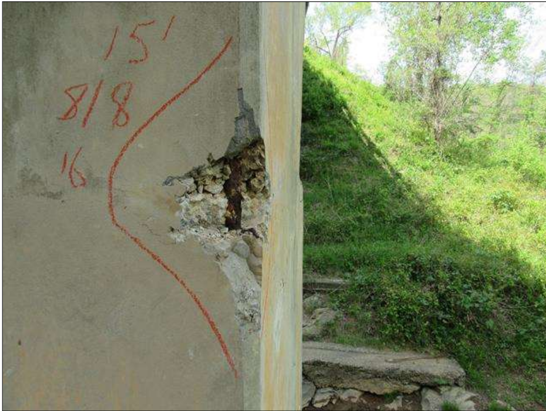
BENT 2 PILE 1 CRACKED SPALL DELAMINATED ON NE CORNER OF PILE 15' ABOVE FOOTING EXTENDS UP 16" & 8" ON EACH FACE.
