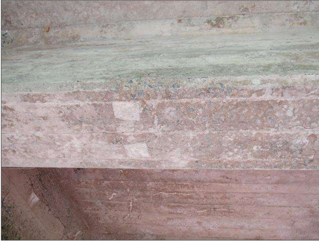
Span 5 Beam 4: 15 Feet of Cracking (RC and Other): Width 0.012-0.05 in. or spacing of 1.0-3.0 ft. SPAN 5 BOTTOM OF BEAM 5 HAS SCATTERED MAP CRACKS AND LONGITUDINAL CRACKS ALONG THE BOTTOM FROM BENT 4 OUT.
