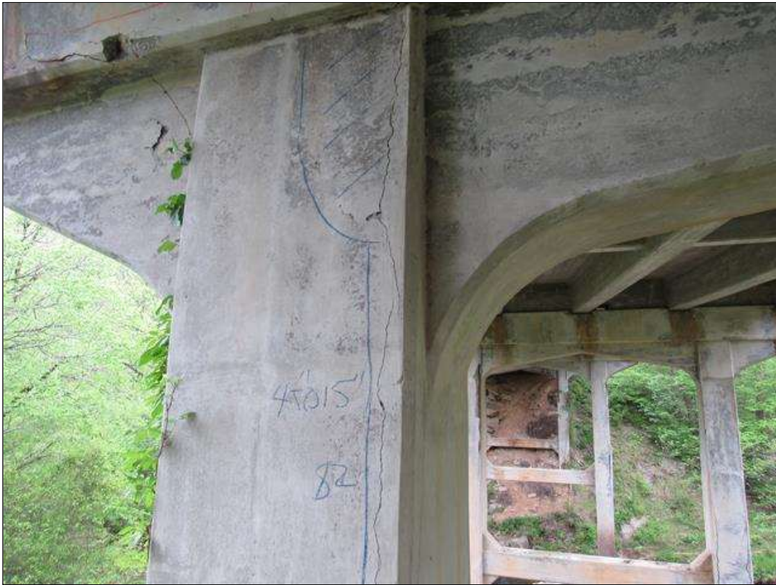
Bent 1 Pile 1: 1 Each of Delamination/Spall/Patched Area: Delaminated. Spall 1 in. or less deep or 6 in. or less in diameter. Patched area that is sound. BENT 1 PILE 1 SOUTH WEST CORNER OF PILE HAS CRACKED DELAMINATED AREA FROM TOP DOWN 82". 4 TO 15" ON WEST FACE AN 4" ON SOUTH FACE.
