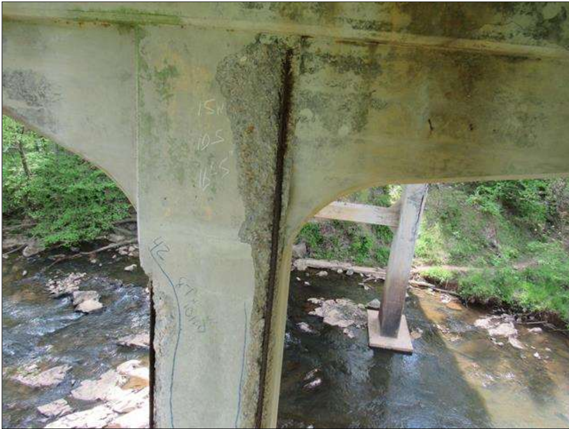
Bent 2 Pile 1: 0 Each of Delamination/Spall/Patched Area: Spall greater than 1 in. deep or greater than 6 in. diameter. Patched area that is unsound or showing distress. Does not warrant structural review. BENT 2 PILE 1 HAS A CRACKED SPALL DELAMINATED AREA ON SW CORNER FM BOTTOM OF CAP DOWN 16' 5" FROM 8 TO 15 ON WEST FACE AND 10" ON SOUTH. LARGE REBAR EXPOSED.
