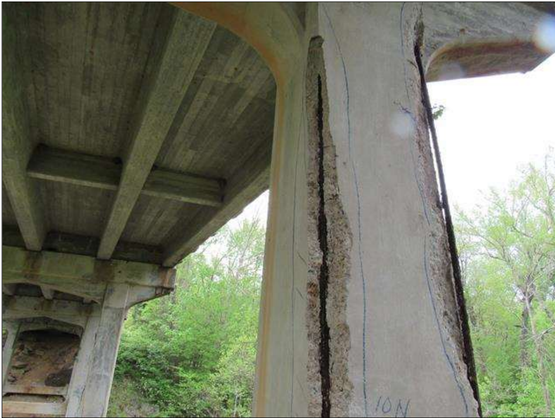
Bent 1 Pile 2: 0 Each of Delamination/Spall/Patched Area: Spall greater than 1 in. deep or greater than 6 in. diameter. Patched area that is unsound or showing distress. Does not warrant structural review. BENT 1 PILE 2 CRACKED DELAMINATED SPALL AREA ON NW CORNER OF PILE STARTS 35" BELOW CAP EXTENDS DOWN 8' 10" ON NORTH FACE 8" ON WEST.
