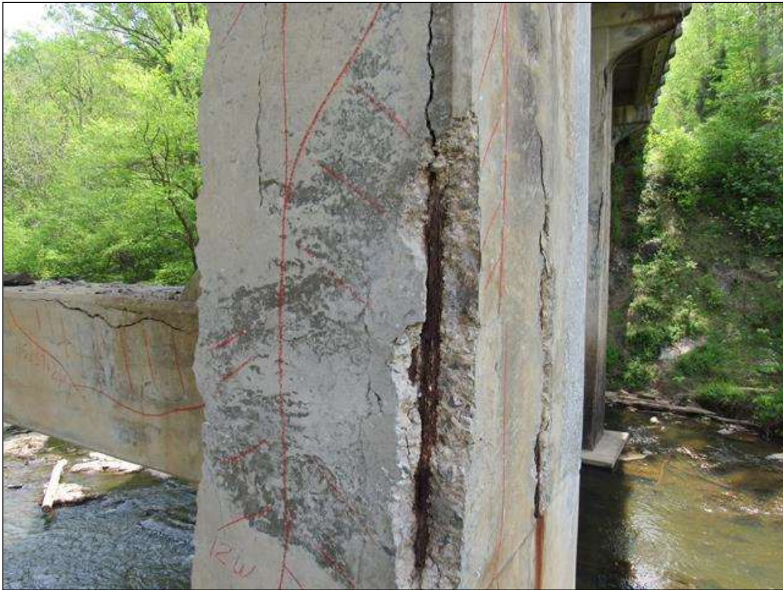
BNT 2 PILE 2 CRACKED SPALL DELAM AREA SW CORNER STARTS 14' ABOVE FOOTING EXTEND UP 8' 4" FM 6" TO 16' ON WEST FACE AND 10" ON SOUTH WITH REBAR EXPOSED
