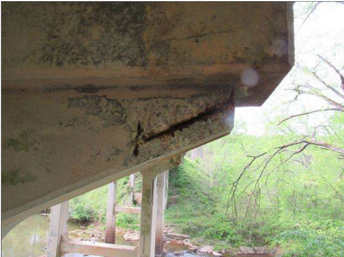
BENT 5 EAST FACE OF HUANCH UNDER LEFT END OF CAP SPALL AREA 9" X 18" X 4" UNDER BOTTOM REBAR AND STIRRUPS EXPOSED.
