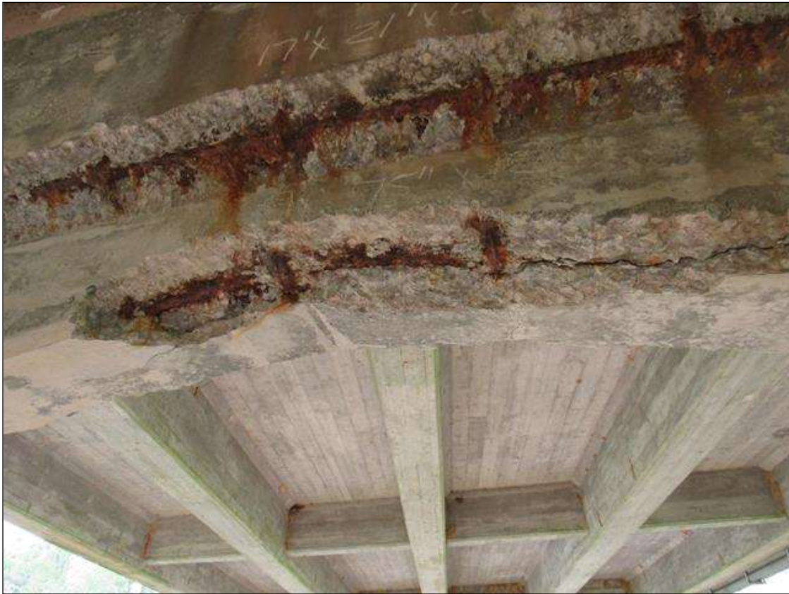
BENT 4 EAST FACE AND BOTTOM OF HUANCH UNDER G3 CRACKED SPALL AND DELAMINATED 9" WIDE 75" LONG 6" UNDER BOTTOM WITH REBAR AND STIRRUPS EXPOSED.
