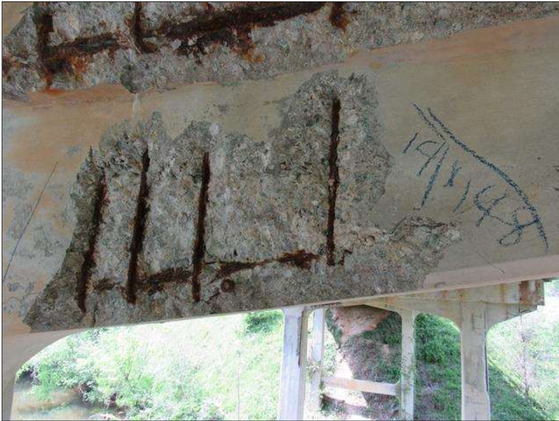
BENT 3 EAST FACE OF HAUNCH UNDER BOTTOM OF CAP SPALL DELAMINATED 19" HIGH 48" LONG 2" DEEP WITH REBAR AND STIRRUPS EXPOSED.
