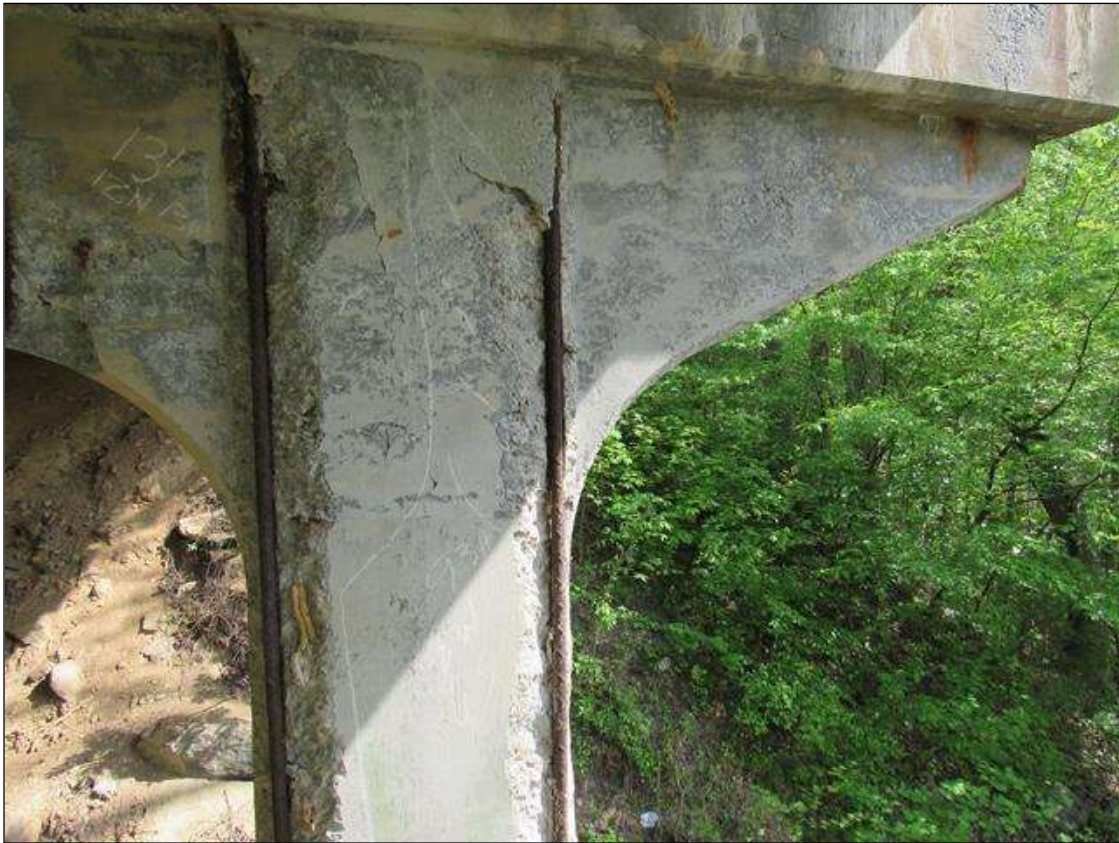
BENT 4 PILE 2 CRACKED DELAMINATED SPALL AREA SW CORNER OF PILE FM BOTTOM OF CAP DOWN 93". 8" ON WEST FACE AND 6" ON SOUTH.
