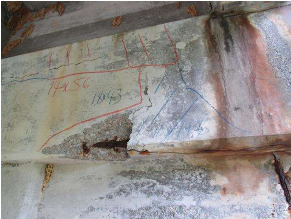
Bent 1 Cap : 0 Feet of Delamination/Spall/Patched Area: Spall greater than 1 inch deep or greater than 6 inches in diameter. Patched area that is unsound or showing distress. Condition does not warrant structural Review BENT 1 EAST OF CAP HAS CRACKED SPALL DELAMINATED AREA ALONG BOTTOM OF CAP RIGHT SIDE OF G1 18" UP FACE 43" LONG SPALL IS 10" X 19" X 6" WITH LARGE REBAR EXPOSED.
