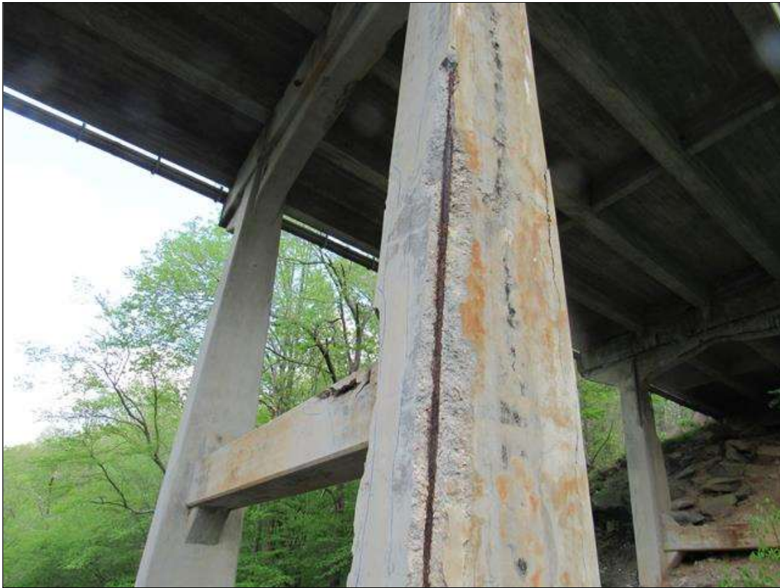
Bent 3 Pile 2: 0 Each of Delamination/Spall/Patched Area: Spall greater than 1 in. deep or greater than 6 in. diameter. Patched area that is unsound or showing distress. Does not warrant structural review. BENT 3 PILE 2 CRACKED SPALL DELAMINATED AREA SW CORNER OF PILE STARTS 32" FM BOTTOM OF CAP EXTENDS DOWN 24' 16" ON WEST FACE 13" ON SOUTH FACE WITH LARGE REAR EXPOSED.
