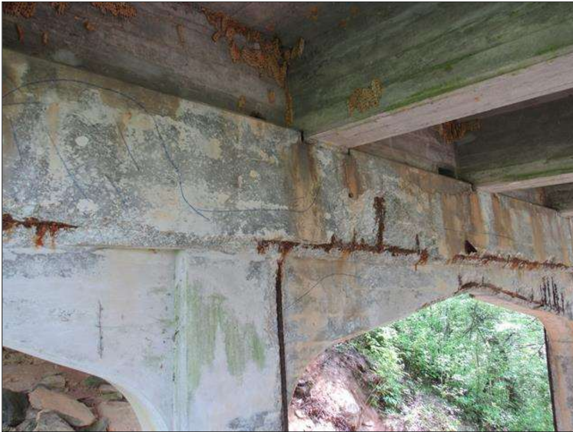
Bent 4 Cap : 27 Feet of Delamination/Spall/Patched Area: Spall greater than 1 inch deep or greater than 6 inches in diameter. Patched area that is unsound or showing distress. Condition does not warrant structural Review BENT 4 WEST FACE OF CAP FM LT END OVER TO PILE 2 CRACKED SPALL DELAMINATED 27' LONG FM 12' TO 30" FM BOTTOM OF CAP UP WITH REBAR AND STIRRUPS EXPOSED.
