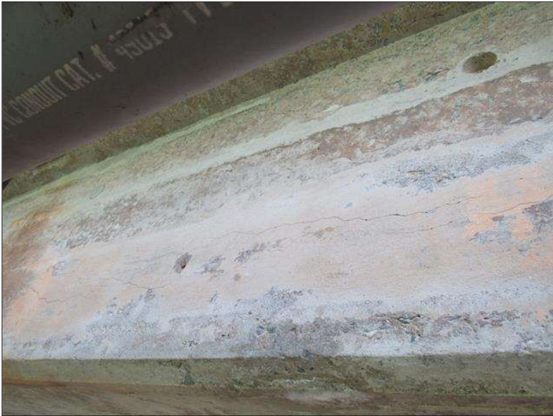
Span 5 Beam 1: 15 Feet of Cracking (RC and Other): Width 0.012-0.05 in. or spacing of 1.0-3.0 ft. SPAN 5 G1 SCATTERED LONGITUDINAL CRACK AND MAP CRACKS.
