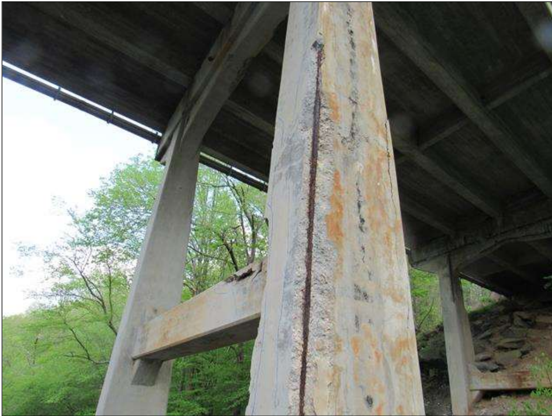
BENT 3 PILE 2 CRCKED SPALL DELAM AREA SW CORNR OF PILE STARTS 32" FM BOTM OF CAP EXTENDS DOWN 24' 16" ON WST FACE 13" ON SOUTH FACE WITH LRG REBAR EXP
