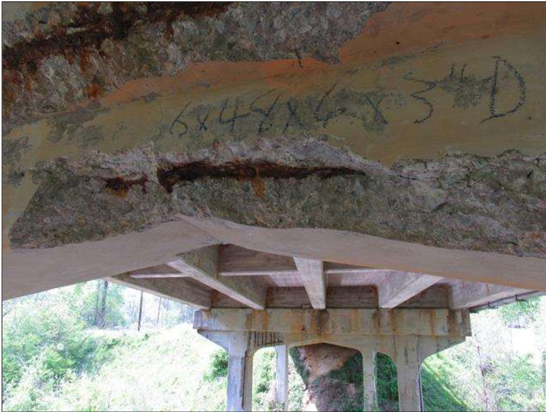
BENT 3 EAST FACE OF HAUNCH UNDER G3 SPALL AND DELAMINATED 6" HIGH 48" LONG 6" UNDER BOTTOM REBAR AND STIRRUPS EXPOSED.
