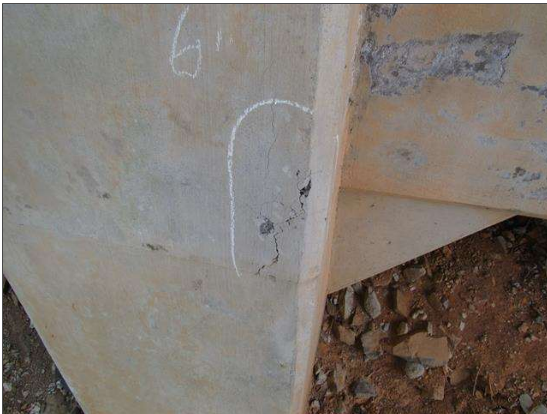
Bent 4 Pile 1: 0 Each of Delamination/Spall/Patched Area: Delaminated. Spall 1 in. or less deep or 6 in. or less in diameter. Patched area that is sound. BENT 4 PILE 1 CRACKED DELAMINATED ON SW CORNER STARTS 3' ABOVE GROUND LINE 12 HIGH AND 6" ON EACH FACE.
