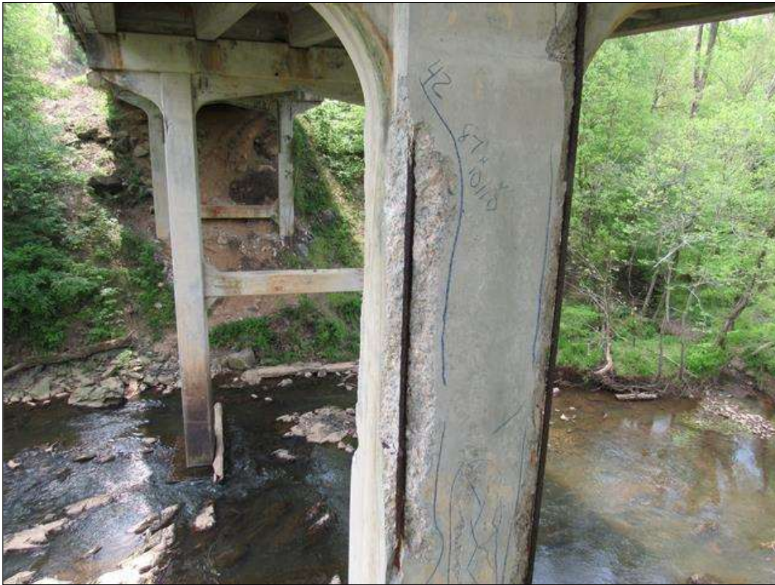
Bent 2 Pile 1: 1 Each of Delamination/Spall/Patched Area: Spall greater than 1 in. deep or greater than 6 in. diameter. Patched area that is unsound or showing distress. Does not warrant structural review. BENT 2 PILE 1 CRACKED SPALL DELAMINATED AREA NW CORNER OF PILE STARTS 42" BELOW CAP EXTENDS DOWN 87" AND 10" ON EACH FACE.
