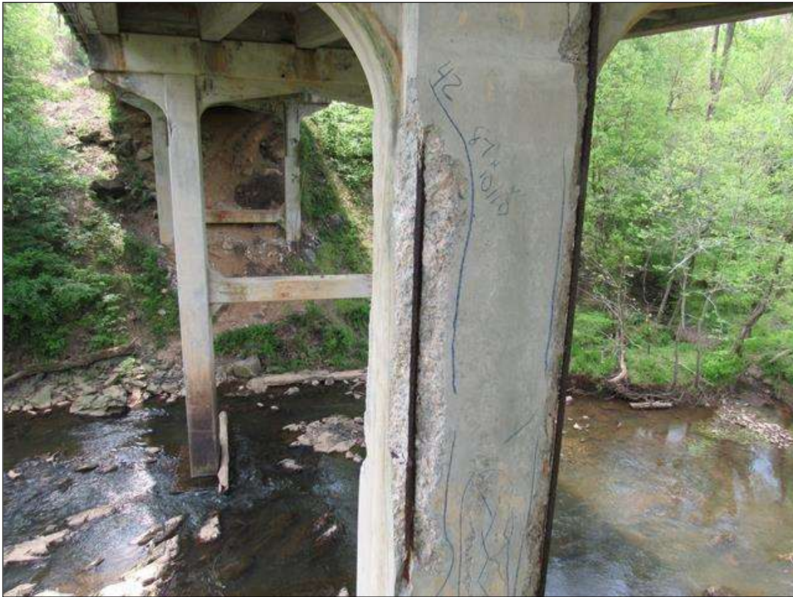
BENT 2 PILE 1 CRACKED SPALL DELAMINATED AREA NW CORNER OF PILE STARTS 42" BELOW CAP EXTENDS DOWN 87" AND 10" ON EACH FACE.
