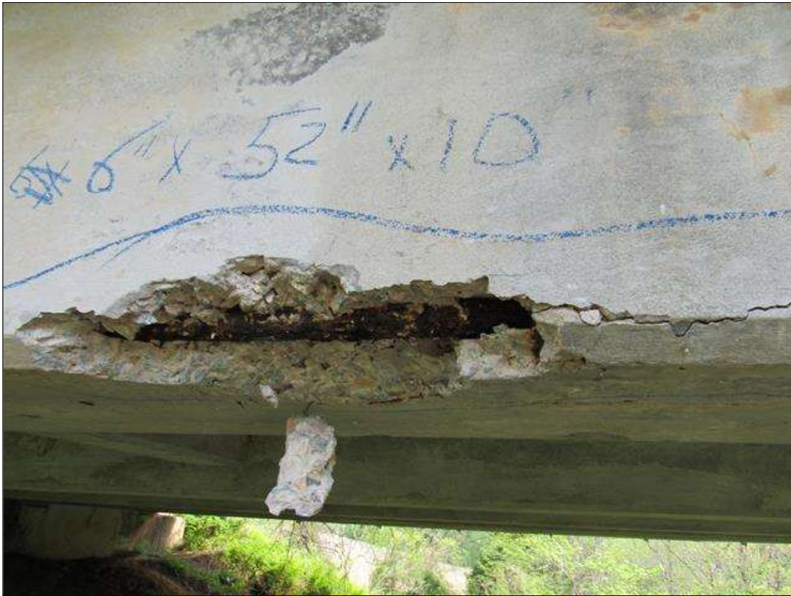
Span 1 Beam 5: 5 Feet of Delamination/Spall/Patched Area: Spall greater than 1 in. deep or greater than 6 in. diameter. Patched area that is unsound or showing distress. Does not warrant structural review. SPAN 1 GIRDER 5 HAS A CRACKED SPALL DELAMINATED AREA LOCATED AT 15' FM BENT 1. 6" UP FACE 52" LONG 10" UNDER BOTTOM WITH LARGE REBAR EXPOSED.
