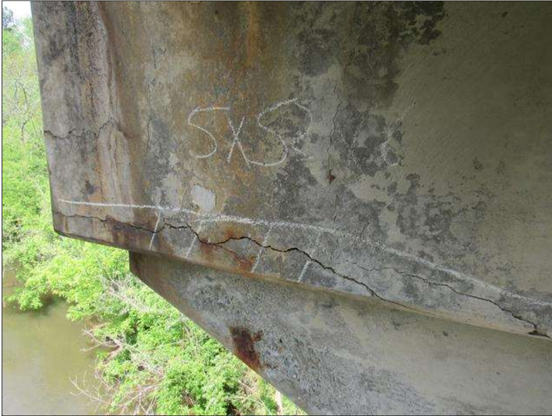
Bent 2 Cap : 5 Feet of Delamination/Spall/Patched Area: Delaminated. Spall 1 inch or less deep or 6 inches or less in diameter. Patched area that is sound BENT 2 EAST FACE OF CAP HAS A CRACKED DELAMINATED AREA ALONG THE BOTTOM EDGE 5" UP FACE 52" LONG 6" UNDER BOTTOM.
