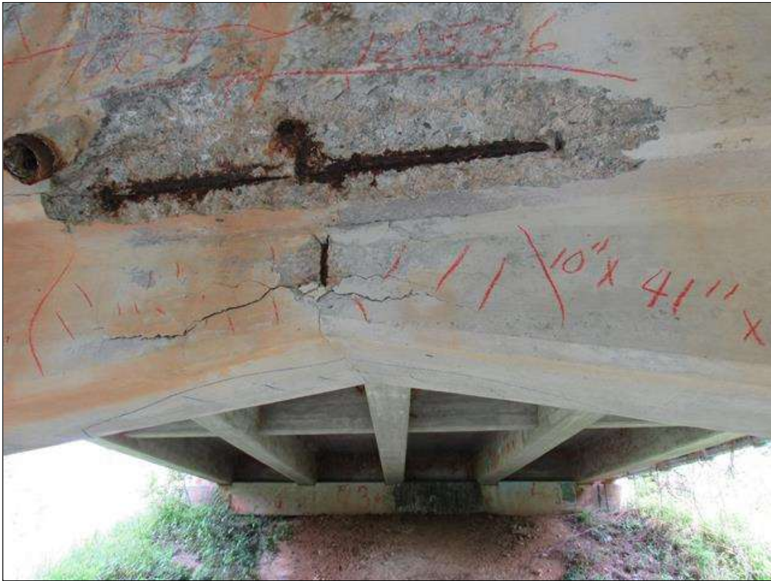
HAUNCH AREA UNDER BENT 1 CAP UNDER GIRDER 3 CRACKED AND DELAMINATED WITH A 6" X 6" X 3/4" SPALL AREA.
