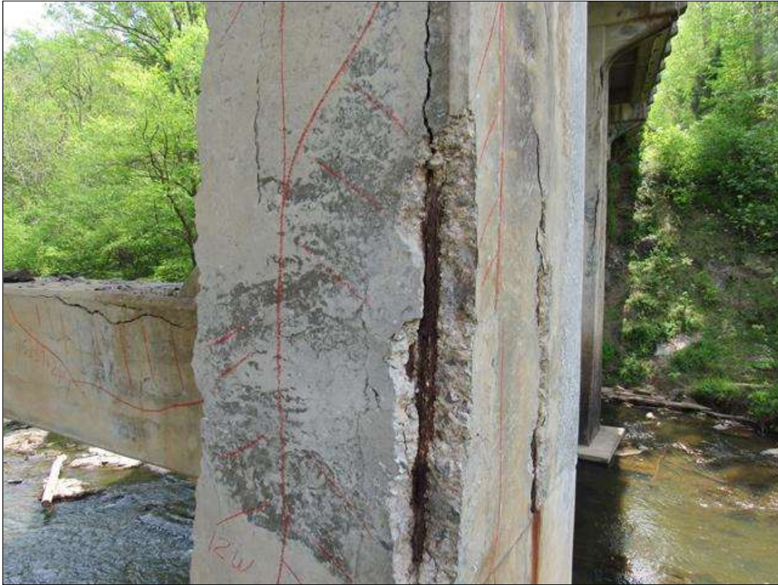
Bent 2 Pile 2: 0 Each of Delamination/Spall/Patched Area: Spall greater than 1 in. deep or greater than 6 in. diameter. Patched area that is unsound or showing distress. Does not warrant structural review. BENT 2 PILE 2 CRACKED SPALL DELAMINATED AREA SW CORNER STARTS 14' ABOVE FOOTING EXTENDS UP 8' 4" FM 6" TO 16' ON WEST FACE AND 10" ON SOUTH. REBAR EXPOSED.
