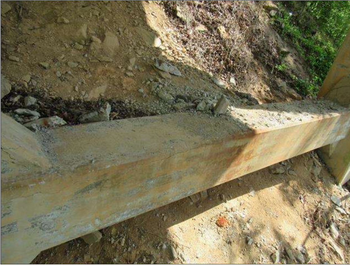
BENT 4 HORZ STRUT BETWEEN PILES 1 AND 2 IS CRACKED AND DELAMINATED 24" ON TOP 8" DOWN FACE ALL THE WAY ACROSS.
