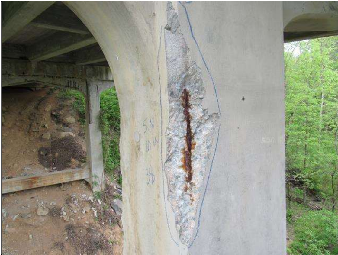
Bent 3 Pile 1: 1 Each of Delamination/Spall/Patched Area: Spall greater than 1 in. deep or greater than 6 in. diameter. Patched area that is unsound or showing distress. Does not warrant structural review. BENT 3 NW CORNER OF PILE 1 SPALL AREA 33" BELOW CAP EXTENDS DOWN 38". 5" ON NORTH 10" ON WEST WITH LARGE REBAR EXPOSED.
