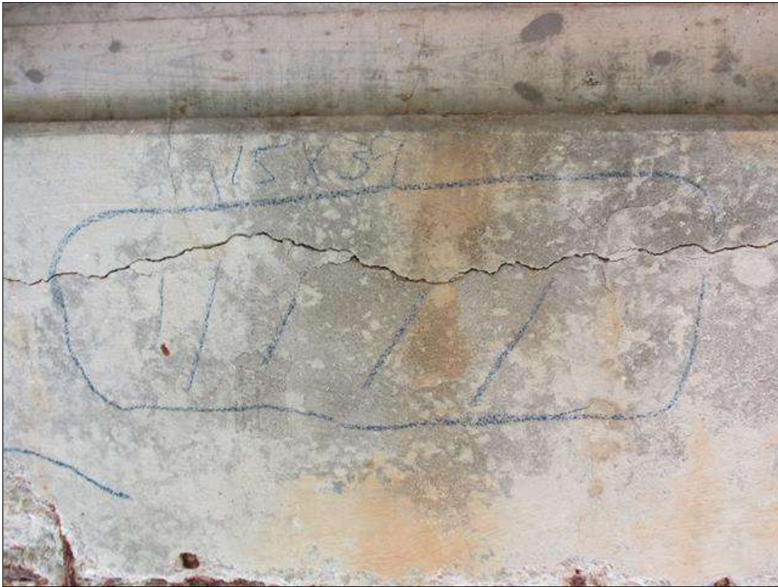
Bent 3 Cap : 0 Feet of Delamination/Spall/Patched Area: Delaminated. Spall 1 inch or less deep or 6 inches or less in diameter. Patched area that is sound BENT 3 EAST OF CAP HAS A CRACKED AND DELAMINATED AREA BETWEEN GIRDERS 3 AND 4. 15" X 39".
