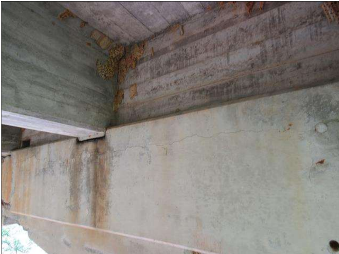
Bent 3 Cap : 0 Feet of Cracking (RC and Other); Width 0.012-0.05 in. or spacing of 1.0-3.0 ft. BENT 3 EAST FACE OF CAP HAS A HORZ CRACK FROM G1 TO G5 10" TO 12" DOWN FACE.
