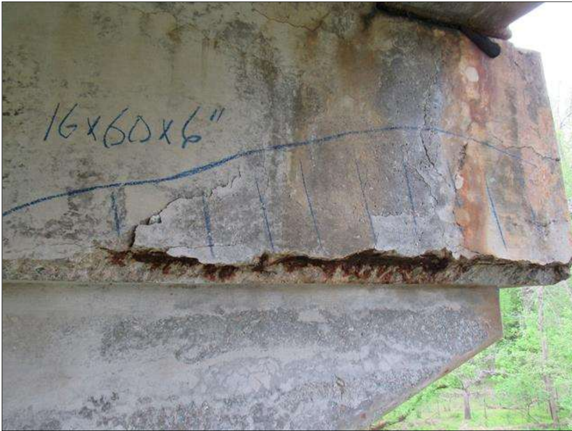
Bent 1 Cap : 0 Feet of Delamination/Spall/Patched Area: Spall greater than 1 inch deep or greater than 6 inches in diameter. Patched area that is unsound or showing distress. Condition does not warrant structural Review BENT 1 WEST FACE OF CAP CRACKED SPALL DELAMINATED AREA FM RIGHT END BACK 60" 16" UP FACE 6" UNDER BOTTOM WITH REBAR AND STIRRUPS EXPOSED.
