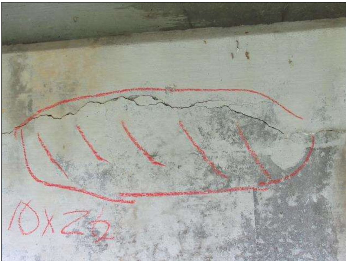
Bent 1 Cap : 2 Feet of Delamination/Spall/Patched Area: Delaminated. Spall 1 inch or less deep or 6 inches or less in diameter. Patched area that is sound. BENT 1 WEST FACE OF CAP HAS A HORZ CRACKED DELAMINATED AREA RIGHT SIDE OF GIRDER 1 THAT IS 10" X 24".
