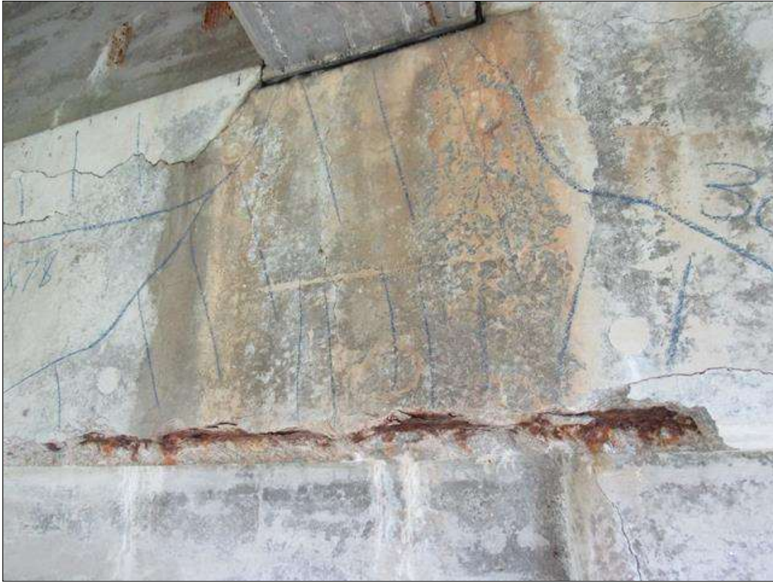
Bent 1 Cap : 0 Feet of Delamination/Spall/Patched Area: Spall greater than 1 inch deep or greater than 6 inches in diameter. Patched area that is unsound or showing distress. Condition does not warrant structural Review BENT 1 WEST FACE OF CAP CRACKED SPALL AND DELAMINATED AREA UNDER G4 TOP DOWN 30" & 78" WIDE 6" UNDER BOTTOM REBAR AND STIRRUPS EXPOSED.
