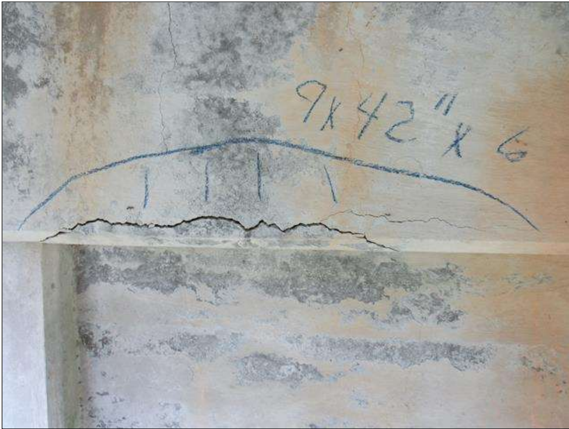
Bent 1 Cap : 0 Feet of Delamination/Spall/Patched Area: Delaminated. Spall 1 inch or less deep or 6 inches or less in diameter. Patched area that is sound BENT EAST FACE OF CAP HAS A CRACKED AND DELAMINATED AREA UNDER GIRDER 4 UNDER BOTTOM EDGE OF CAP.
