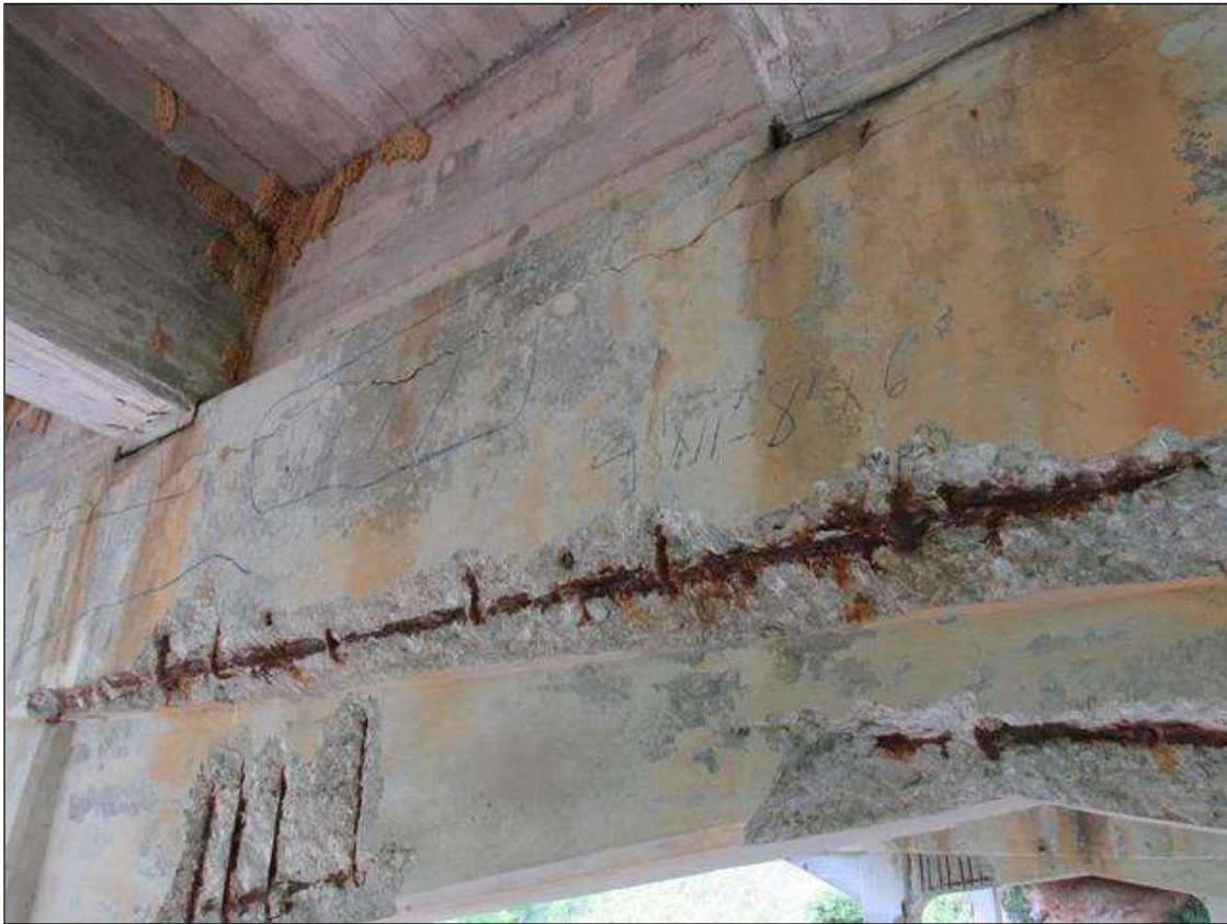
BNT 3 EAST FACE OF CAP HAS A DELAM AND SPALL AREA ALONG BOTM EDGE OF CAP FM G3 TO RT OF G4. 9" UP FACE 11' 8" LONG 6" UNDR BOTM REBAR STIRRUPS EXPOSED
