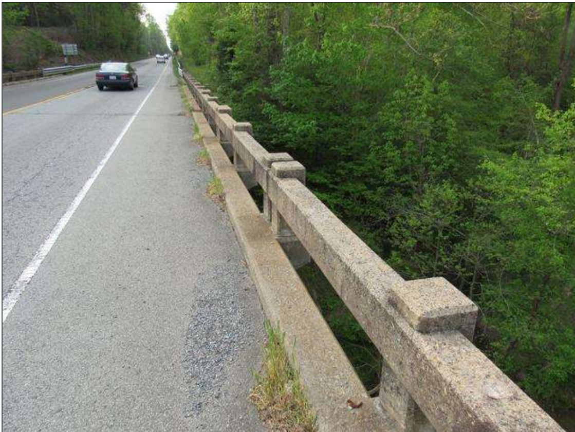
Span 3 Right Bridge Rail: 25 Feet of Cracking (RC and Other): Width 0.012-0.05 in. or spacing of 1.0-3.0 ft. SPAN 3 RIGHT RAIL TOP AND CURB SURFACE SCALING AND MAP CRACKING.
