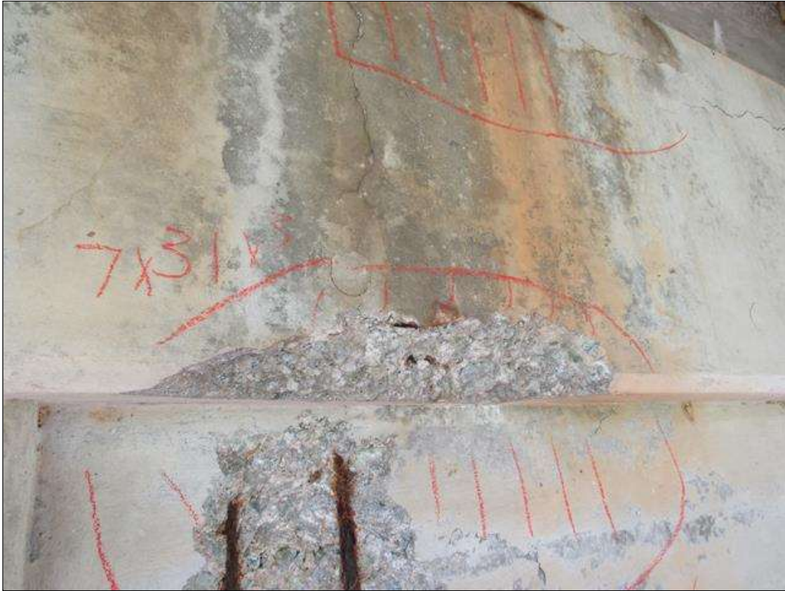
Bent 3 Cap : 3 Feet of Delamination/Spall/Patched Area: Delaminated. Spall 1 inch or less deep or 6 inches or less in diameter. Patched area that is sound BENT 3 WEST FACE OF CAP HAS A SPALL AREA ALONG BOTTOM EDGE UNDER GIRDER 2 7" UP FACE 31" LONG 3" DEEP 6" UNDER BOTTOM.
