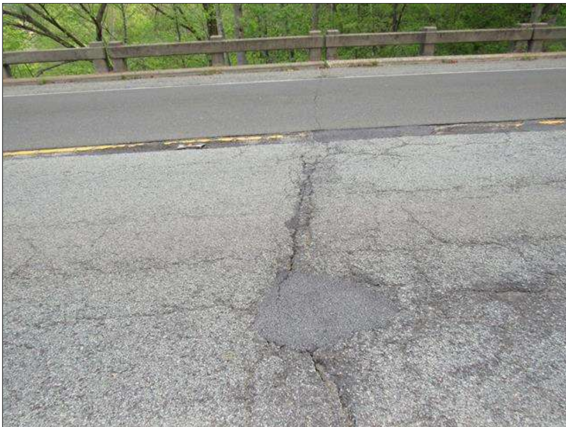
ASPHALT WEARING SURFACE IS CRACKED OVER TOP OF BENT 4. BENG 1, 2, AND 3 ARE SIMILAR.
