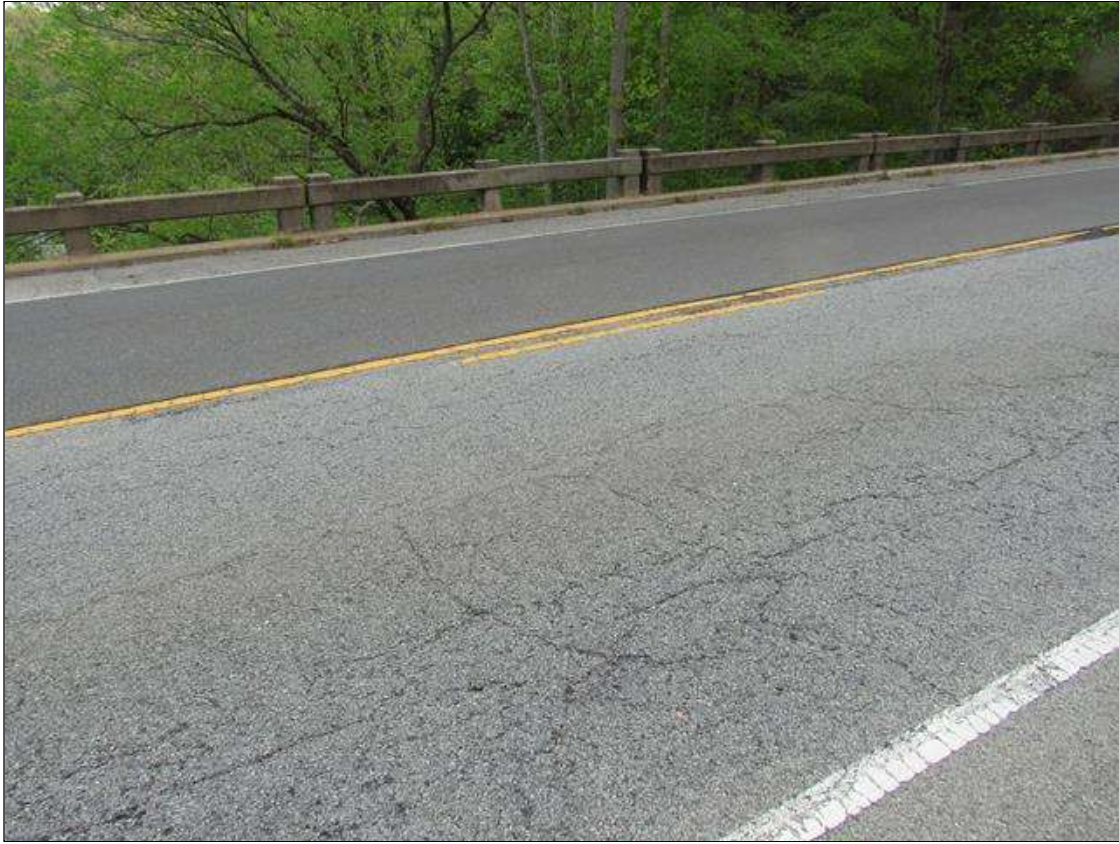
Span 4 Wearing Surface: 1615 Square Feet of Crack (Wearing Surface): Width 0.012-0.05 in. or spacing of 1.0-3.0 ft. SPAN 4 WEARING SURFACE IS HEAVILY MAP CRACKED LEFT AND RIGHT LANE.
