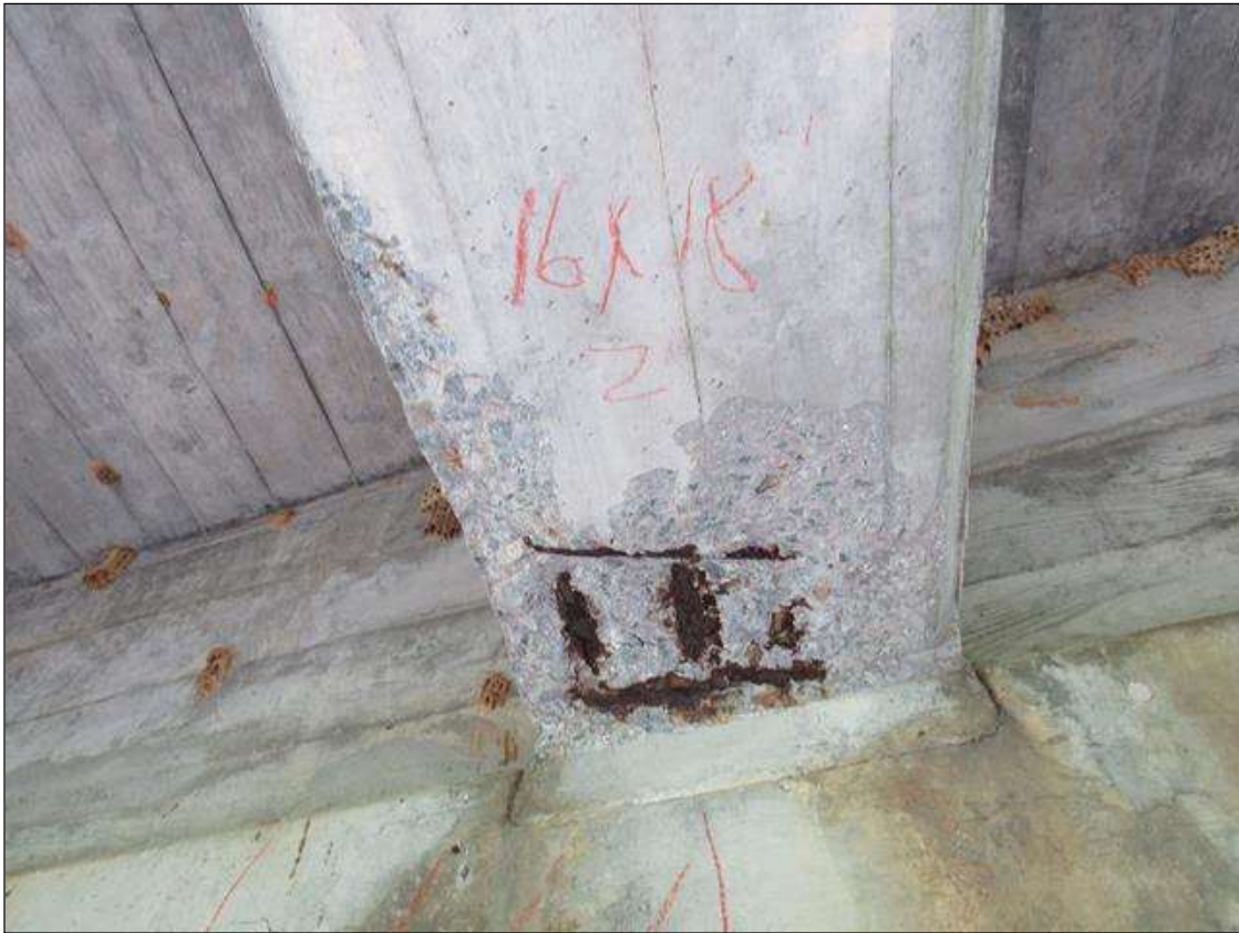
SPAN 3 BEAM 2 AT BENT 2 BOTTOM OF GIRDER HAS A SPALL AREA 16" W FROM CAP OUT 18" AND 2" DEEP REBAR AND STIRRUPS EXPOSED.
