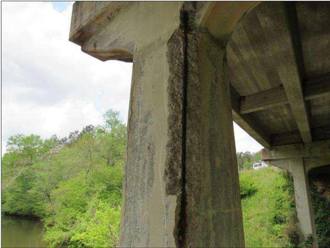
BENT 2 PILE 2 CRACKED DELAMINATED AND SPALL AREA ON NE CORNER OF PILE STARTS 26" BELOW THE CAP EXTENDS DOWN 90" 11" ON EAST FACE AND 8" ON NORTH.
