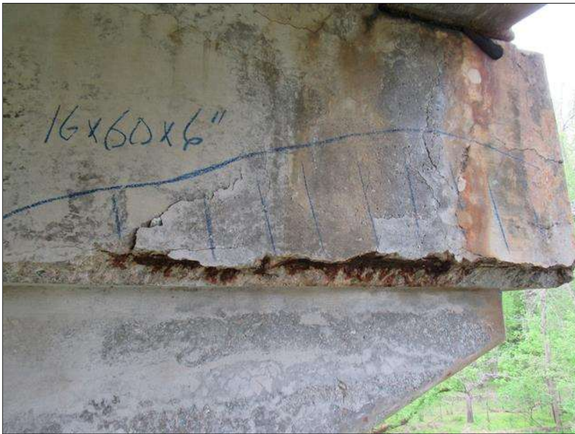
BENT 1 WEST FACE OF CAP CRACKED SPALL DELAMINATED AREA FM RIGHT END BACK 60" 16" UP FACE 6" UNDER BOTTOM WITH REBAR AND STIRRUPS EXPOSED.
