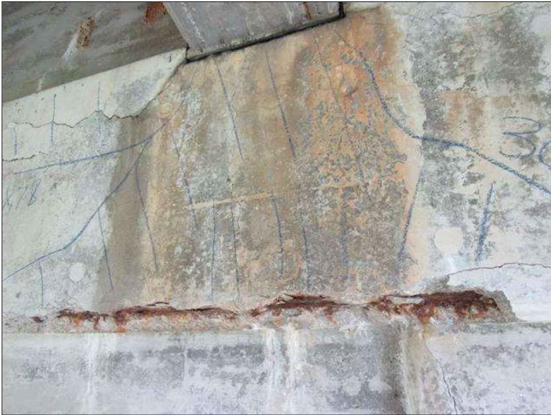
BENT 1 WEST FACE OF CAP CRACKED SPALL AND DELAMINATED AREA UNDER G4 TOP DOWN 30" & 78" WIDE 6" UNDER BOTTOM REBAR AND STIRRUPS EXPOSED.
