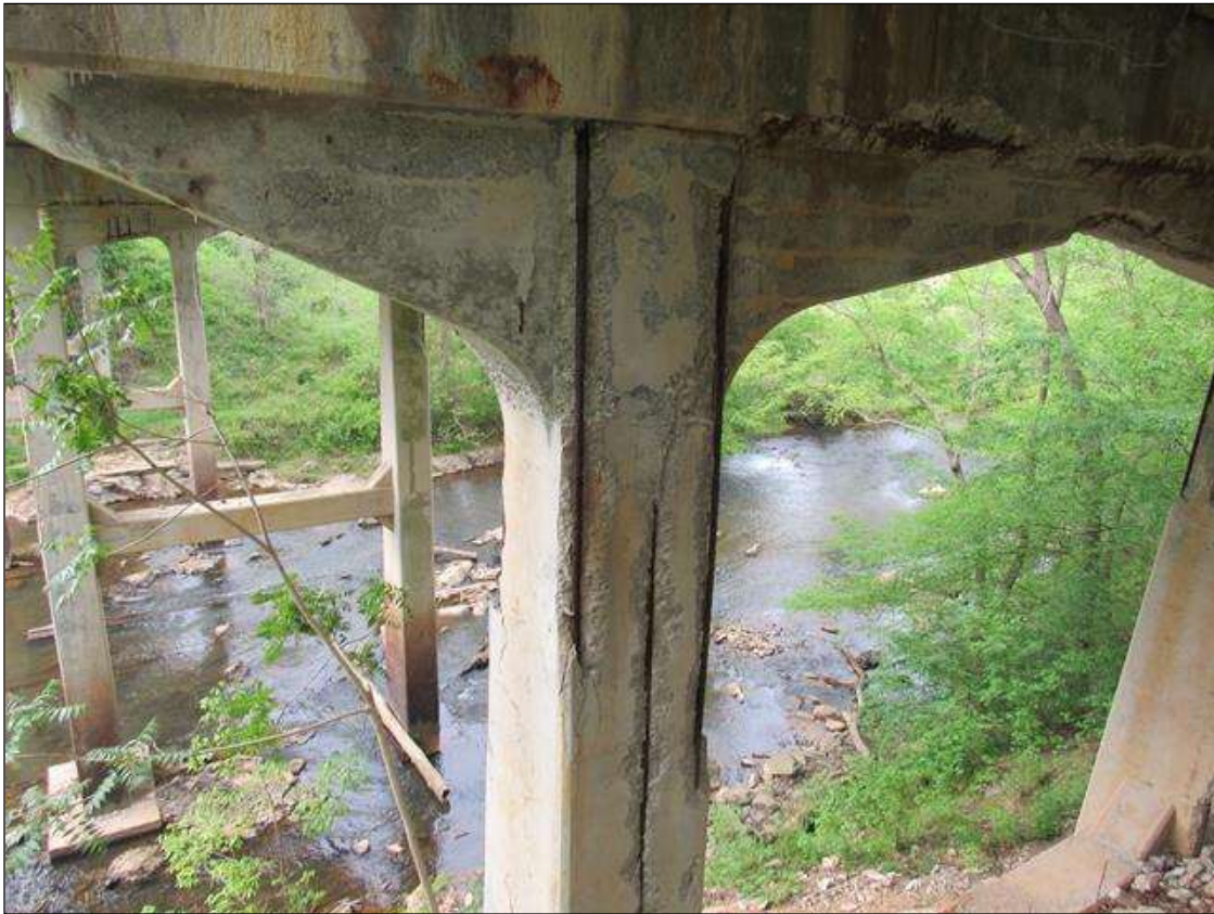
BENT 4 PILE 2 CRACKED SPALL DELAMINATED SE AND NORTH FACE FM CAP DOWN 13' & 32" WIDE ON EAST FACE & 6" ON SOUTH AND NORTH.
