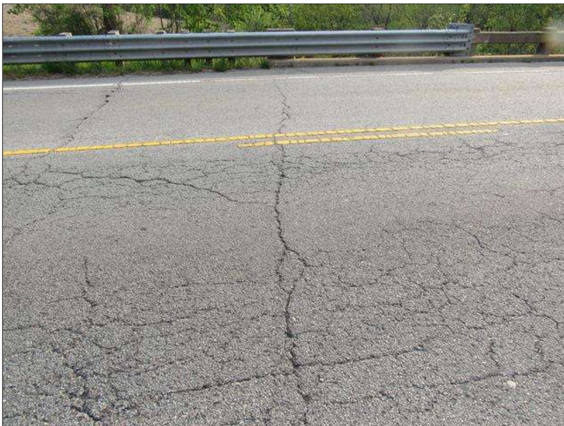
ASPHALT WEARING SURFACE OVER END BENT 1 CRACKED WITH END BENT 2 SIMILAR.
