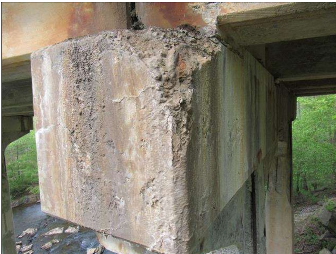
Bent 4 Cap : 0 Feet of Delamination/Spall/Patched Area: Delaminated. Spall 1 inch or less deep or 6 inches or less in diameter. Patched area that is sound BENT 4 RIGHT END OF CAP HEAVILY CRACKED WITH EFFLO WITH SPALL AREA IN TOP RIGHT CORNER 12" X 15" X 13" DOWN FACE.
