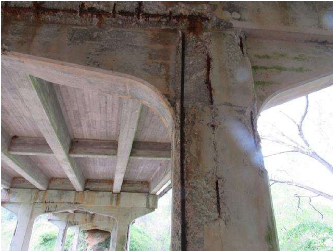
BENT 4 PILE 1 CRACKED SPALL DELAMINATED AREA ON SE CORNER OF PILE FM CAP DOWN 9' 4" AND 10" ON SOUTH 15" ON EAST REBAR EXPOSED.
