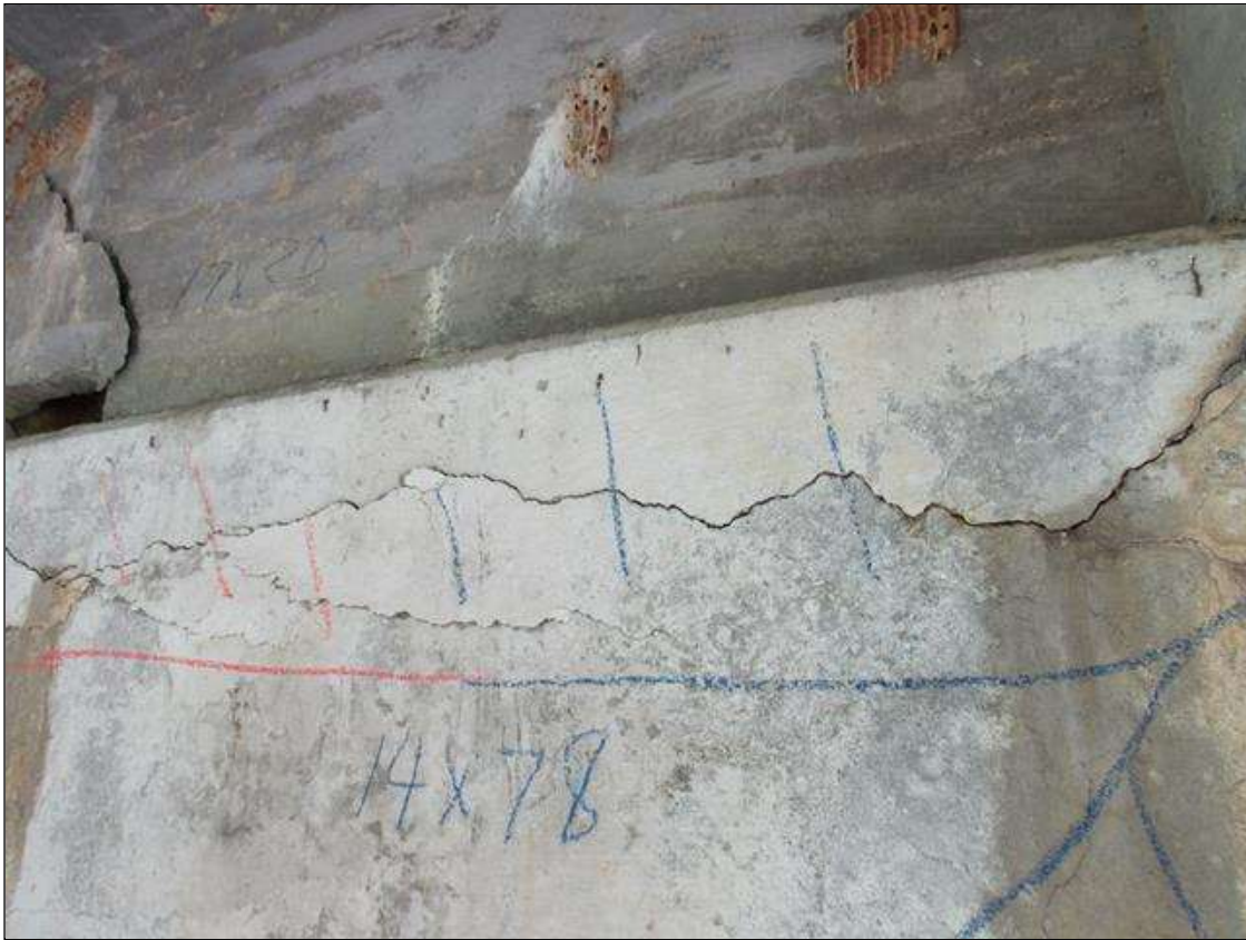
Bent 1 Cap : 6 Feet of Delamination/Spall/Patched Area: Delaminated. Spall 1 inch or less deep or 6 inches or less in diameter. Patched area that is sound BENT 1 WEST FACE OF CAP HAS A CRACKED AND DELAMINATED AREA ALONG TOP EDGE BETWEEN GIRDERS 3 AND 4. 14" DOWN FACE AND 78" LONG.
