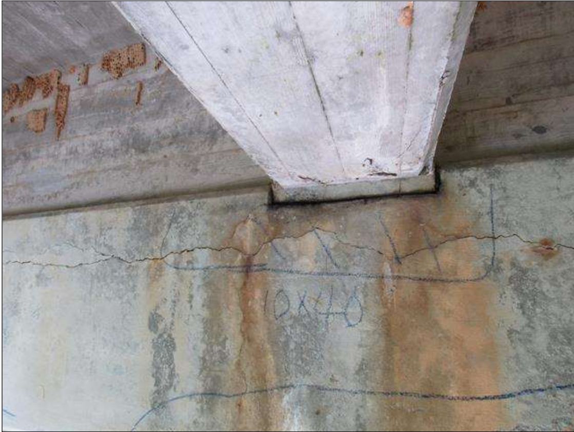
Bent 3 Cap : 0 Feet of Delamination/Spall/Patched Area: Delaminated. Spall 1 inch or less deep or 6 inches or less in diameter. Patched area that is sound BENT 3 EAST FACE OF CAP HAS A HORZ CRACK AND DELAMINATED AREA UNDER GIRDER 4 FROM TOP DOWN 10" AND 40" LONG.
