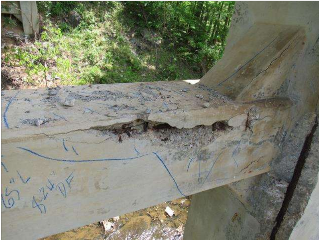
BENT 3 HORZ STRUT AREA LEFT SIDE OF PILE 2 IS CRACKED SPALL DELAMINATED 24" ON TOP 65" LONG AND FROM 8" TO 24" DOWN FACE REBAR AND STIRRUPS EXPOSED.
