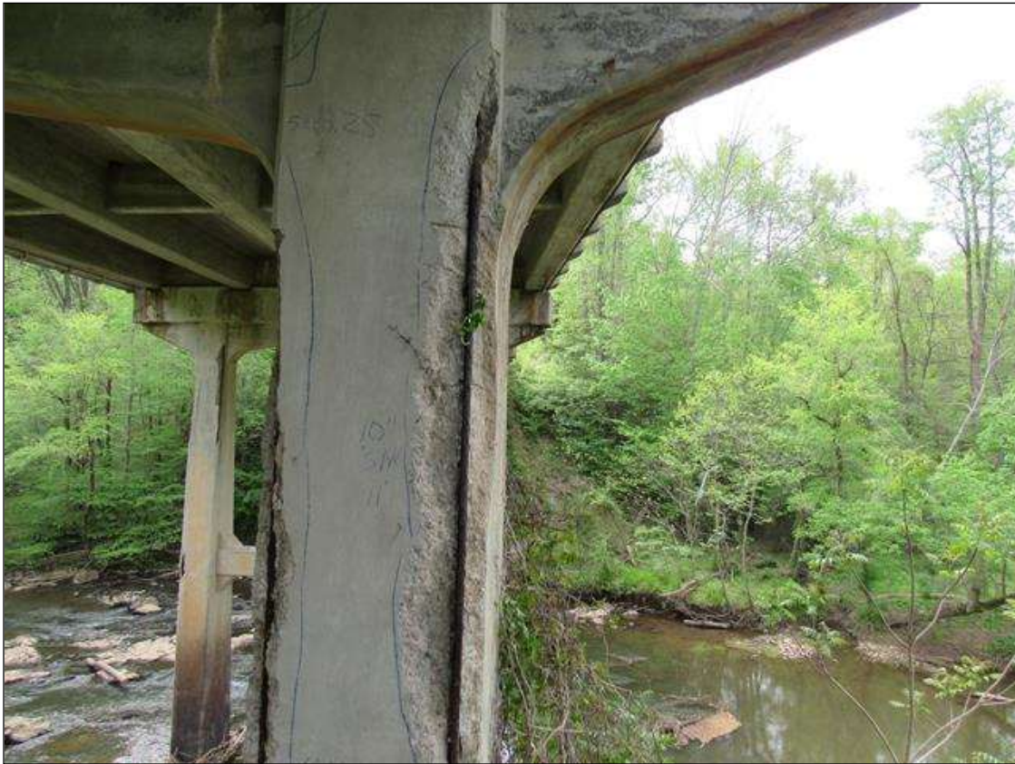
BENT 1 PILE 2 CRCKED DELAM SPALL AREA ON SW CRNER STARTS 20" BELOW BOTTOM OF CAP & EXTENDS DWN 11' & 10" ON SOUTH AND WEST FACE WITH LRGE REBAR EXPOSE
