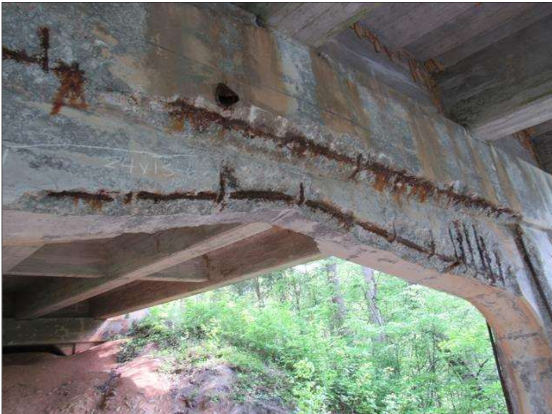
BENT 4 WEST FACE OF HAUNCH CRACKED SPALL DELAMINATED FM 15" TO 24" HIGH 13' 6" LONG 12" UNDER BOTTOM REBAR AND STIRRUPS EXPOSED.
