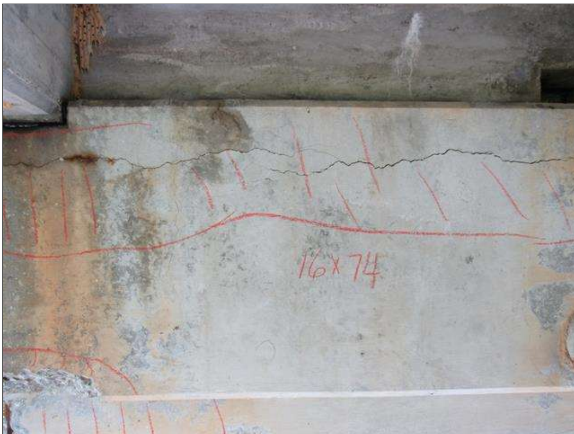
Bent 3 Cap : 7 Feet of Delamination/Spall/Patched Area: Delaminated. Spall 1 inch or less deep or 6 inches or less in diameter. Patched area that is sound BENT 3 EAST FACE OF CAP HORZ CRACK AND DELAMINATED AREA ALONG TOP EDGE OF CAP FROM TOP DOWN 16" AND 74" LONG.
