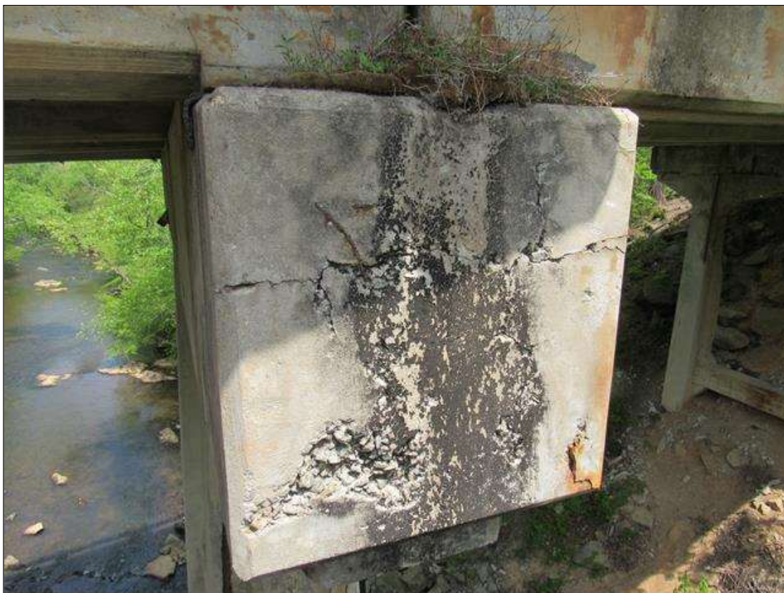
Bent 3 Cap : 0 Feet of Cracking (RC and Other): Width 0.012-0.05 in. or spacing of 1.0-3.0 ft. BENT 3 RIGHT END OF CAP MAP CRACKING AND HAS A 7" X 12" SPALL 1" DEEP.
