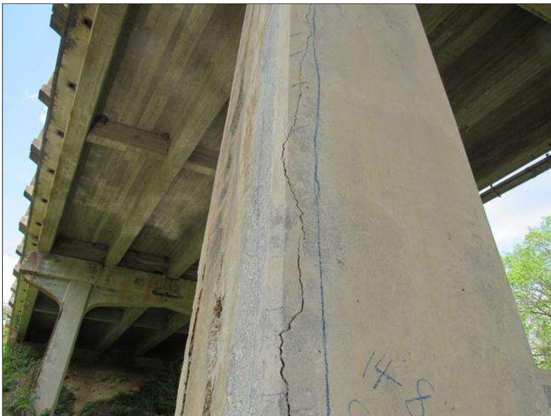
Bent 2 Pile 2: 0 Each of Delamination/Spall/Patched Area: Delaminated. Spall 1 in. or less deep or 6 in. or less in diameter. Patched area that is sound. BENT 2 PILE 2 IS CRACKED AND DELAMINATED ON SE CORNER OF PILE STARTS 14' 8" ABOVE FOOTING EXTENDS UP 94" . 5" ON SOUTH AND EAST FACE.
