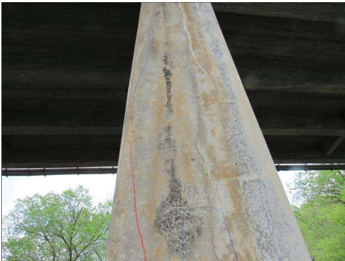
Bent 2 Pile 2: 0 Each of Cracking (RC and Other): Width 0.012-0.05 in. or spacing or 1.0-3.0 ft. BENT 2 PILE 2 HAS VERTICAL CRACKS ON THE FACE OF THE PILE.
