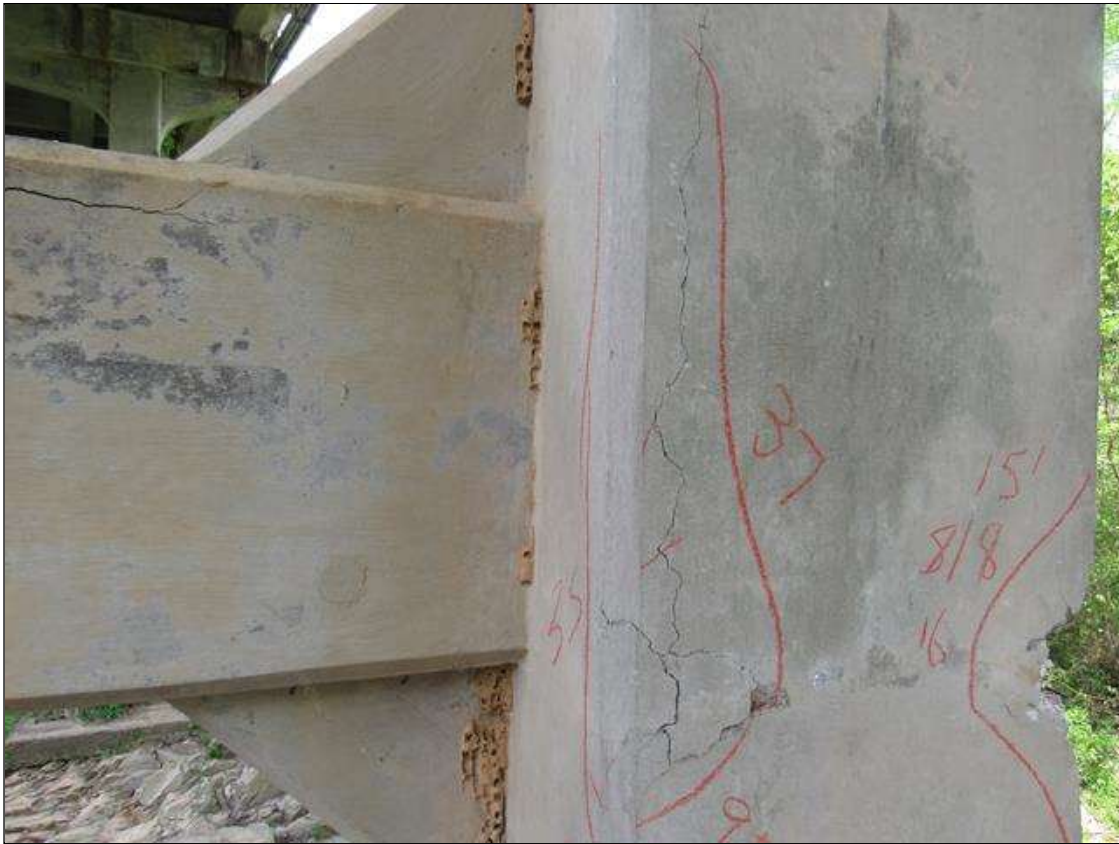
Bent 2 Pile 1: 0 Each of Delamination/Spall/Patched Area: Delaminated. Spall 1 in. or less deep or 6 in. or less in diameter. Patched area that is sound. BENT 2 PILE 1 CRACKED DELAMINATED AREA ON SE CORNER OF PILE AT THE STRUT 3" ON SOUTH FACE 9" ON EAST FACE AND 37" HIGH.
