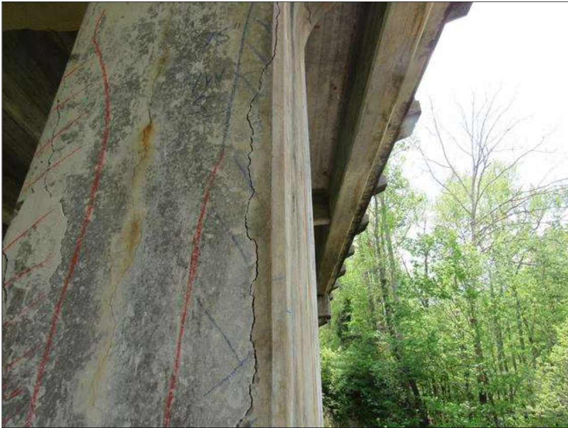
Bent 2 Pile 2: 0 Each of Delamination/Spall/Patched Area: Delaminated. Spall 1 in. or less deep or 6 in. or less in diameter. Patched area that is sound. BENT 2 PILE 2 HAS CRACKED DELAMINATED AREA SW CORNER OF PILE STARTS 53" BELOW CAP EXTENDS DOWN 75". 9" ON WEST FACE AND 5" ON SOUTH.
