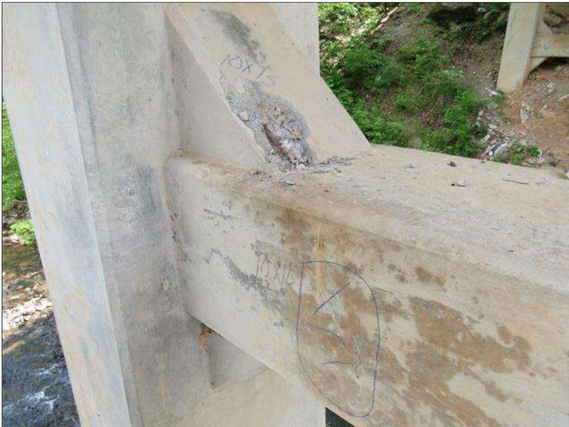
BENT 3 STRUT AREA RIGHT SIDE OF PILE 1 ON TOP AND EAST FACE HAS A 10" X 15" SPALL AREA 1 1/4" DEEP REBAR EXPOSED AND A 10" X 16" CRACKED AND DELAMINATED AREA.
