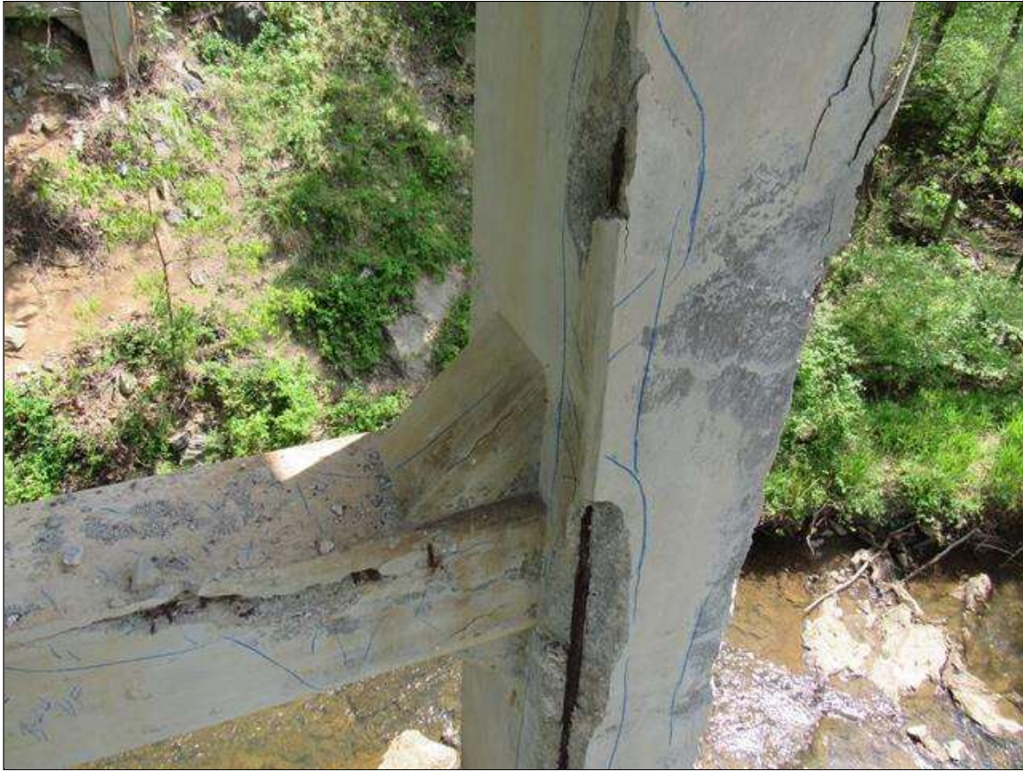
Bent 3 Pile 2: 0 Each of Delamination/Spall/Patched Area: Spall greater than 1 in. deep or greater than 6 in. diameter. Patched area that is unsound or showing distress. Does not warrant structural review. BENT 3 PILE 2 CRACKED SPALL DELAMINATED AREA NW CORNER STARTS 12' ABOVE FOOTING EXTENDS UP 11' 6". 16" ON NORTH AND 11" ON WEST.
