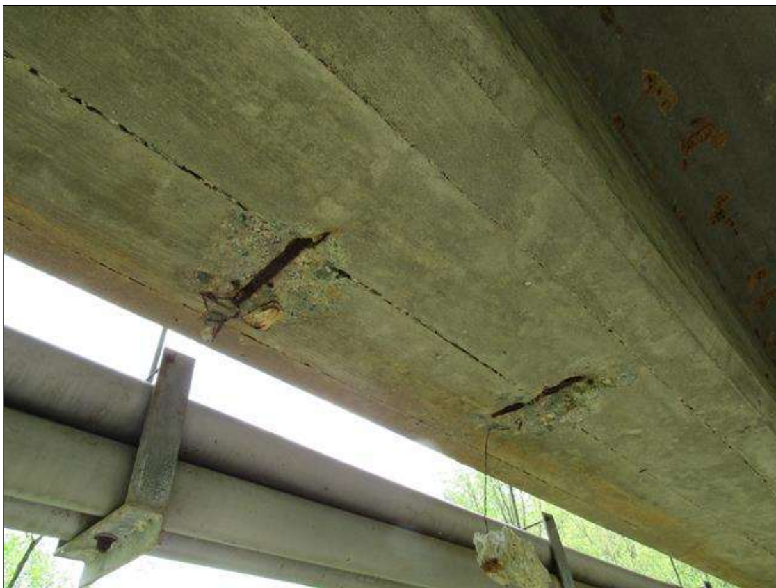
Span 2 Beam 1: 1 Feet of Delamination/Spall/Patched Area: Delaminated. Spall 1 in. or less deep or 6 in. or less in diameter. Patched area that is sound. SPAN 2 GIRDER 1 HAS 2 SURFACE SPALL AREAS IN BOTTOM OF GIRDER 6" X 6" X 9" BOTH ARE 3/4" DEEP WITH REBAR EXPOSED 8' FROM BENT 2 CAP.
