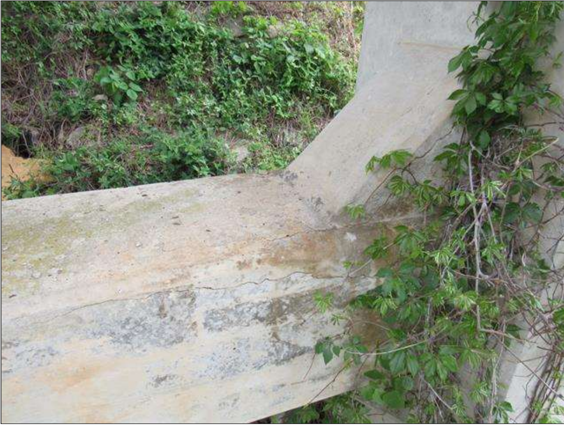
VERTICAL STRUT AT BENT 1 RIGHT SIDE OF PILE 1 CRACKED AND DELAMINATED. 15" ON TOP 5' LONG AND 10" DOWN FACE.
