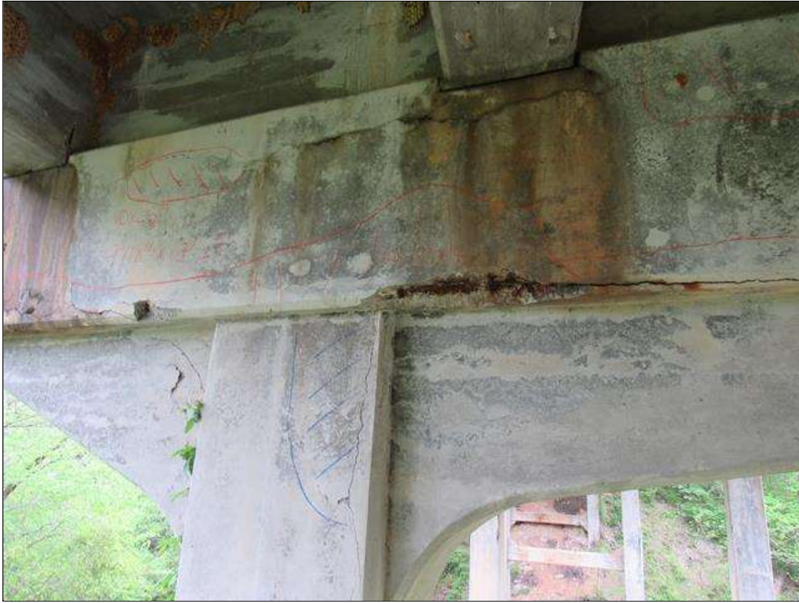
Bent 1 Cap : 13 Feet of Delamination/Spall/Patched Area: Delaminated. Spall 1 inch or less deep or 6 inches or less in diameter. Patched area that is sound BENT 1 WEST FACE OF CAP HAS A CRACKED SPALL DELAMINATED AREA ALONG THE BOTTOM EDGE FM LEFT END TO RIGHT SIDE OF GIRDER 2. 9" TO 18" UP FACE 13' LONG 7" UNDER BOTTOM. SPALL AREA IS 4" X 30" X 4" WITH REBAR EXPOSED.
