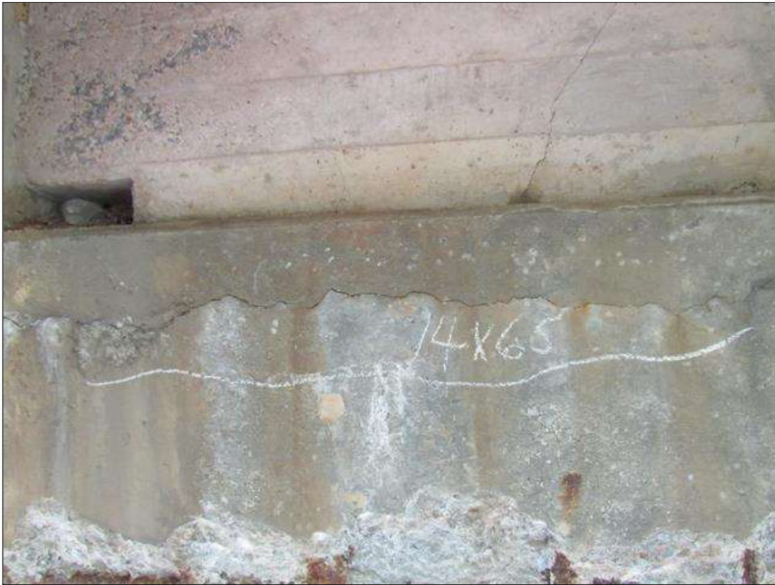
Bent 4 Cap : 0 Feet of Delamination/Spall/Patched Area: Delaminated. Spall 1 inch or less deep or 6 inches or less in diameter. Patched area that is sound BENT 5 EAST FACE OF CAP CRACKED AND DELAMINATED AREAS BETWEEN G2 AND G3 ALONG TOP EDGE. 14" DOWN FACE AND 65" LONG.
