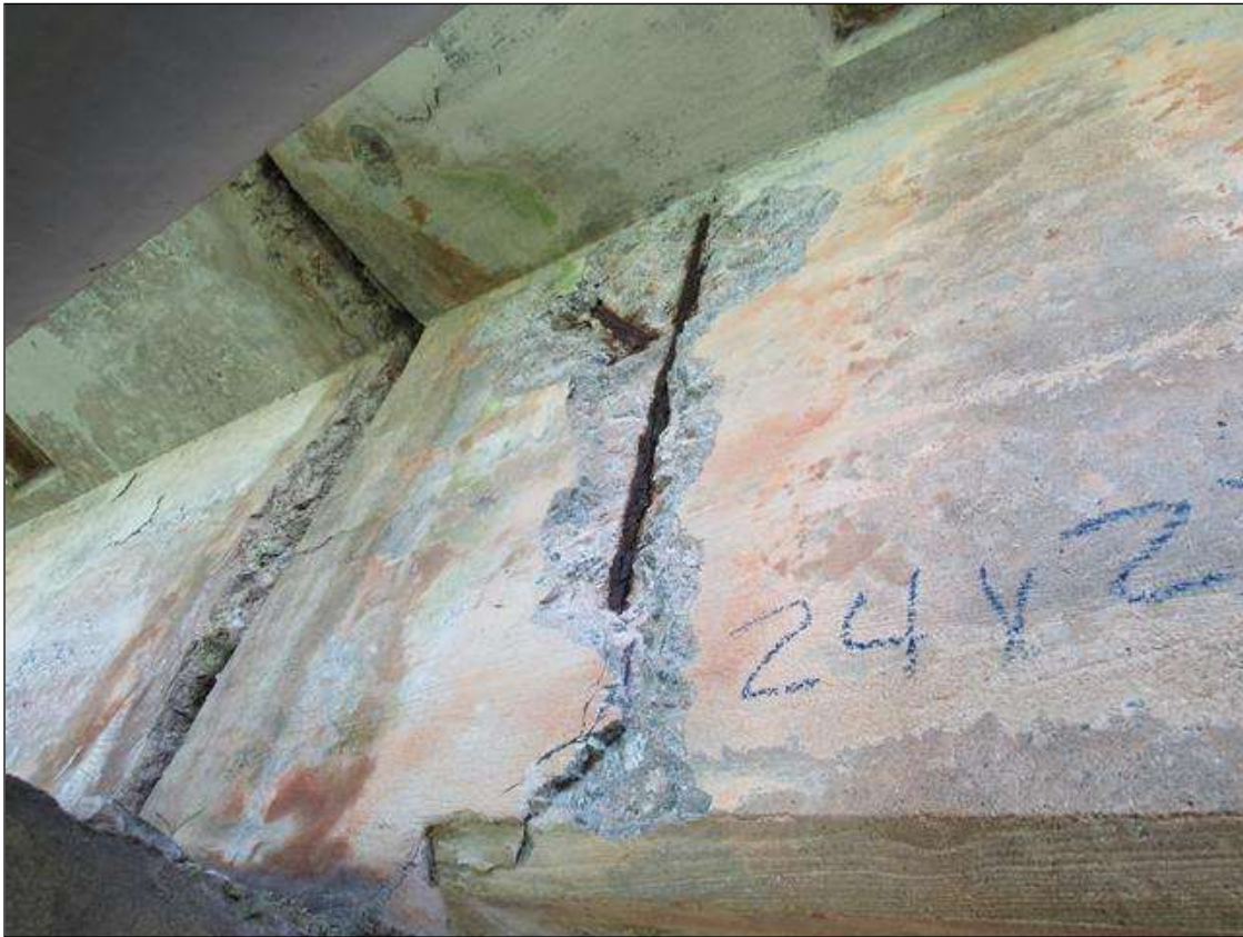
SPAN 4 LEFT SIDE OF G1 OVER BENT 4 CRACKED SPALL DELAMINATED AREA FM END OF GIRDER BACK 24" BOTTOM UP 27" & 1 1/2" DEEP. VERT REBAR EXPOSED.
