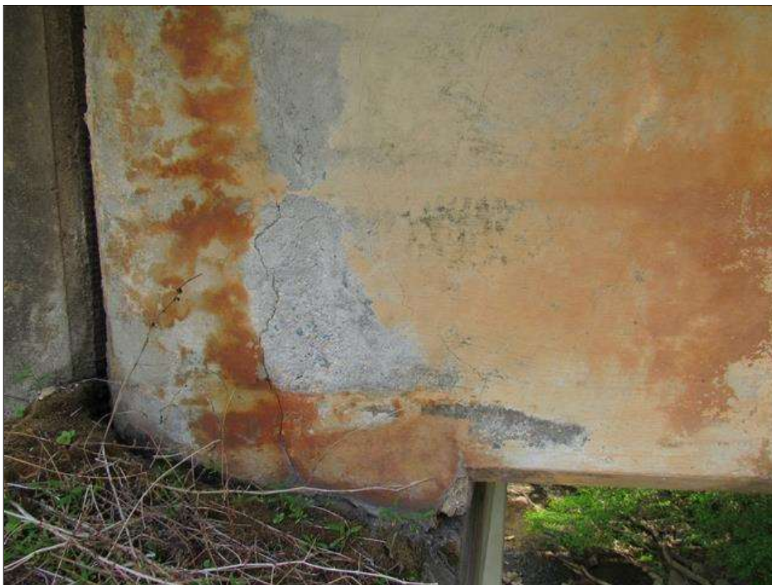
Span 4 Beam 5: 2 Feet of Cracking (RC and Other): Width 0.012-0.05 in. or spacing of 1.0-3.0 ft. SPAN 4 GIRDER 5 CRACKED.
