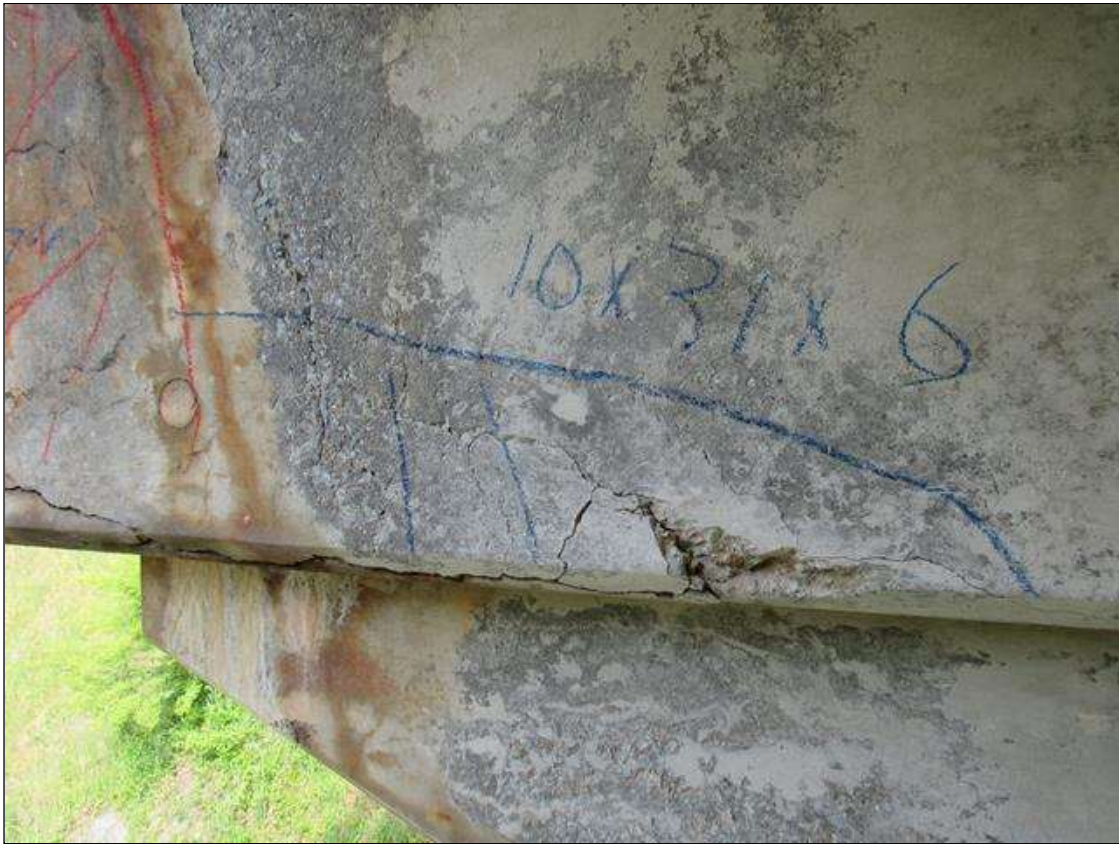
Bent 1 Cap : 0 Feet of Delamination/Spall/Patched Area: Delaminated. Spall 1 inch or less deep or 6 inches or less in diameter. Patched area that is sound BENT 1 EAST FACE OF CAP UNDER GIRDER 5 HAS A CRACKED SPALL DELAMINATED AREA ALONG BOTTOM EDGE 10" UP FACE 31" LONG AND 6" UNDER BOTTOM.
