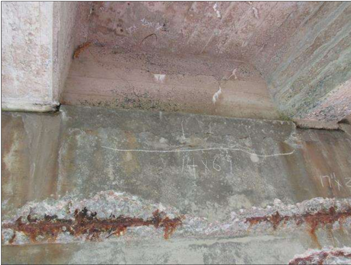
Bent 4 Cap : 0 Feet of Delamination/Spall/Patched Area: Delaminated. Spall 1 inch or less deep or 6 inches or less in diameter. Patched area that is sound BENT 4 EAST FACE OF CAP BETWEEN G3 AND G4 IS CRACKED AND DELAMINATED AREA 14" DOWN FACE AND 67" LONG.
