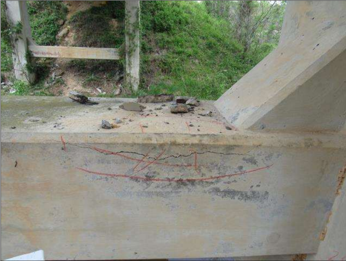
BENT 2 STRUT CRACKED DELAMINATED AREA RIGHT SIDE OF PILE 1 7" DOWN FACE 10" ON TOP 24" LONG. LEFT SIDE OF PILE 2 SIMILAR AREA.
