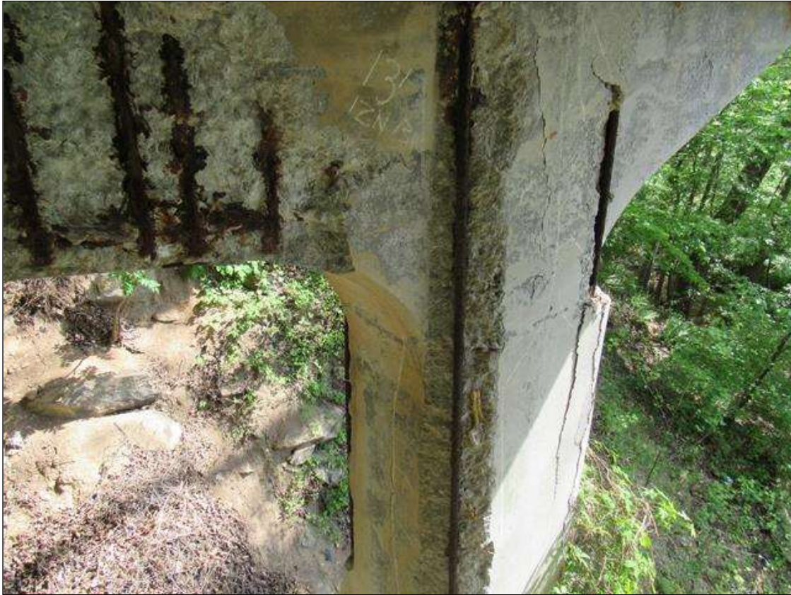
Bent 4 Pile 2: 1 Each of Delamination/Spall/Patched Area: Spall greater than 1 in. deep or greater than 6 in. diameter. Patched area that is unsound or showing distress. Does not warrant structural review. BENT 4 PILE 2 CRACKED SPALL DELAMINATED NW CORNER FM CAP DOWN 13' & 12" ON NORTH FACE 13" ON WEST. REBAR EXPOSED.
