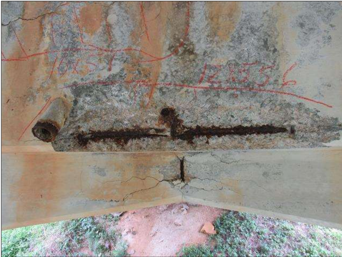
BENT 1 EAST OF CAP HAS CRACKED SPALL DELAM AREA ALONG BOTOM EDGE OF CAP UNDER G 3. 12" UP FACE 15" LONG 6" UNDER BOTTOM REBAR AND STIRRUPS EXPOSED.
