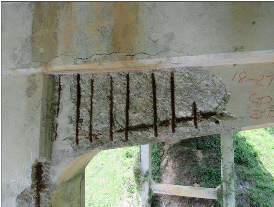
BENT 2 EAST FACE OF HAUNCH UNDER BOTTOM OF CAP LEFT OF PILE 2 CRACKED SPALL AND DELAMINATED. 18" TO 27" DWN FACE 60" LONG 2" D REBAR AND STIRUPS EXPOS
