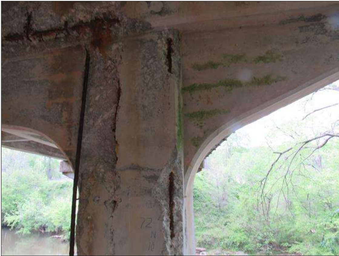
Bent 4 Pile 1: 0 Each of Delamination/Spall/Patched Area: Spall greater than 1 in. deep or greater than 6 in. diameter. Patched area that is unsound or showing distress. Does not warrant structural review. BENT 4 PILE 1 CRACKED SPALL AREA NE CORNER CAP DOWN 72" & 10" ON NORTH FACE & 12" ON EAST WITH REBAR EXPOSED.
