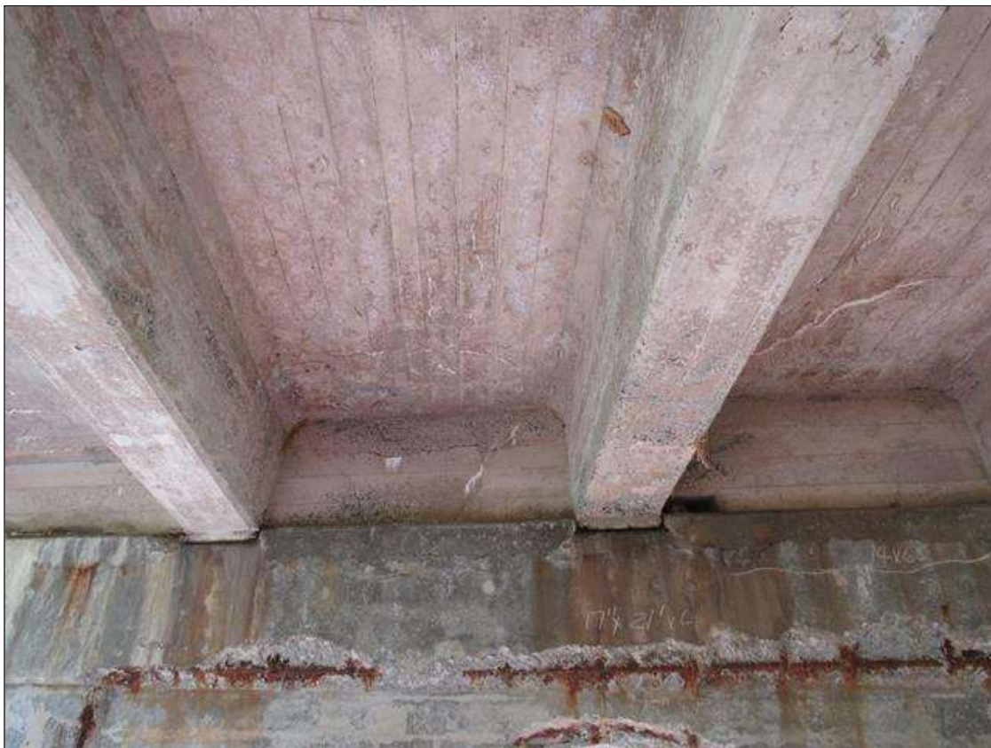
END DIAPHRAGM OVER BENT 4 IN BAYS 2, 3 AND 4 ON EAST FACE ARE CRACKED WITH EFFLO STAINS.
