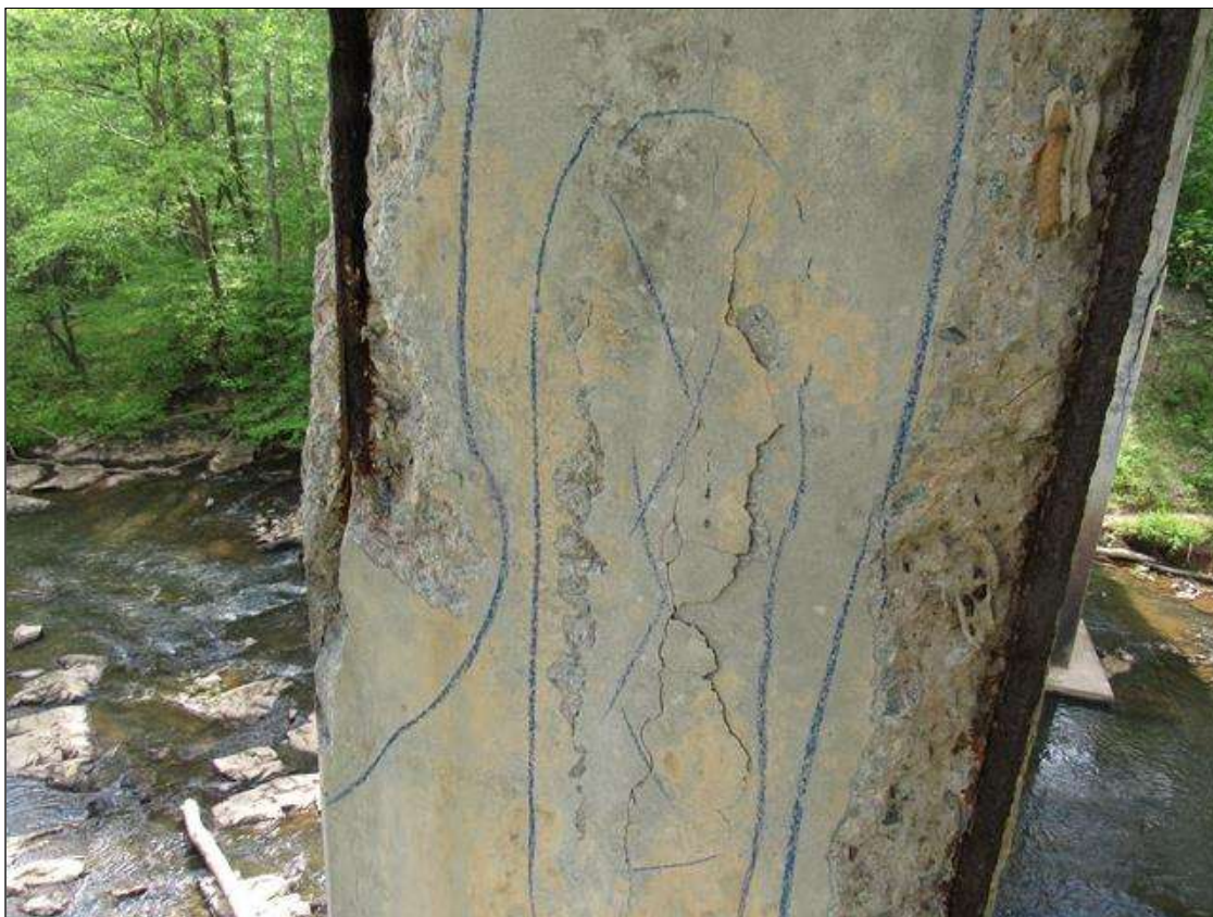
Bent 2 Pile 1: 0 Each of Delamination/Spall/Patched Area: Delaminated. Spall 1 in. or less deep or 6 in. or less in diameter. Patched area that is sound. BENT 2 PILE 1 HAS A CRACKED DELAMINATED AREA ON WEST FACE 100" BELOW BOTTOM OF CAP 9" X 36".
