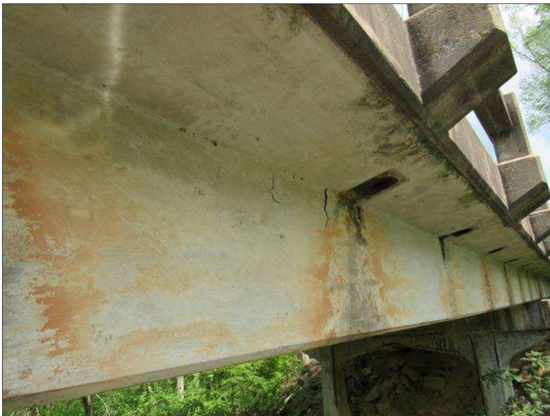
Span 4 Beam 5: 2 Feet of Delamination/Spall/Patched Area: Delaminated. Spall 1 in. or less deep or 6 in. or less in diameter. Patched area that is sound. SPAN 4 GIRDER 5 RIGHT SIDE HAS 3 SURFACE SPALL AREAS NEAR BENT 3 WITH EFFLO STAINS.
