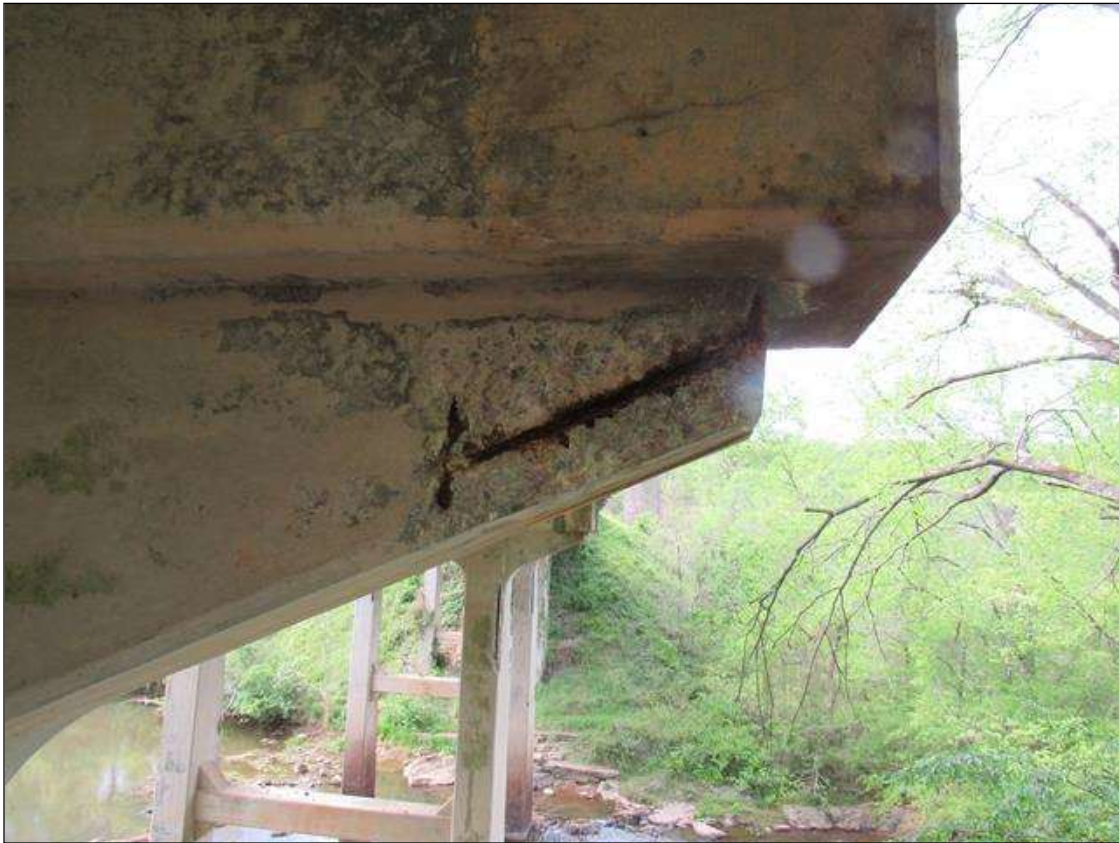
BENT 5 EAST FACE OF HUANCH UNDER LEFT END OF CAP SPALL AREA 9" X 18" X 4" UNDER BOTTOM REBAR AND STIRRUPS EXPOSED.
