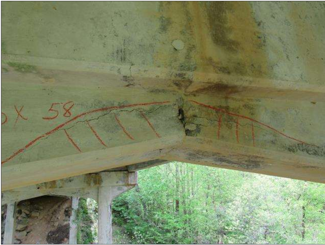
HAUNCH AREA UNDER BOTTOM OF BENT 2 CAP WEST FACE HAS A CRACKED DELAMINATED SPALL AREA. 8" X 58". SPALL AREA IS 8" X 8" X 3/4" DEEP.
