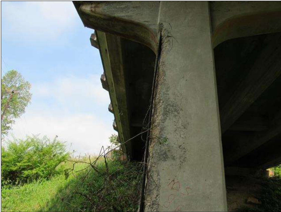
BENT 1 PILE 2 CRACKED SPALL DELAMINATED ON SE CORNER OF PILE 10" ON SOUTH FACE 8" ON EAST 11" DOWN FACE START 32" BELOW THE CAP.
