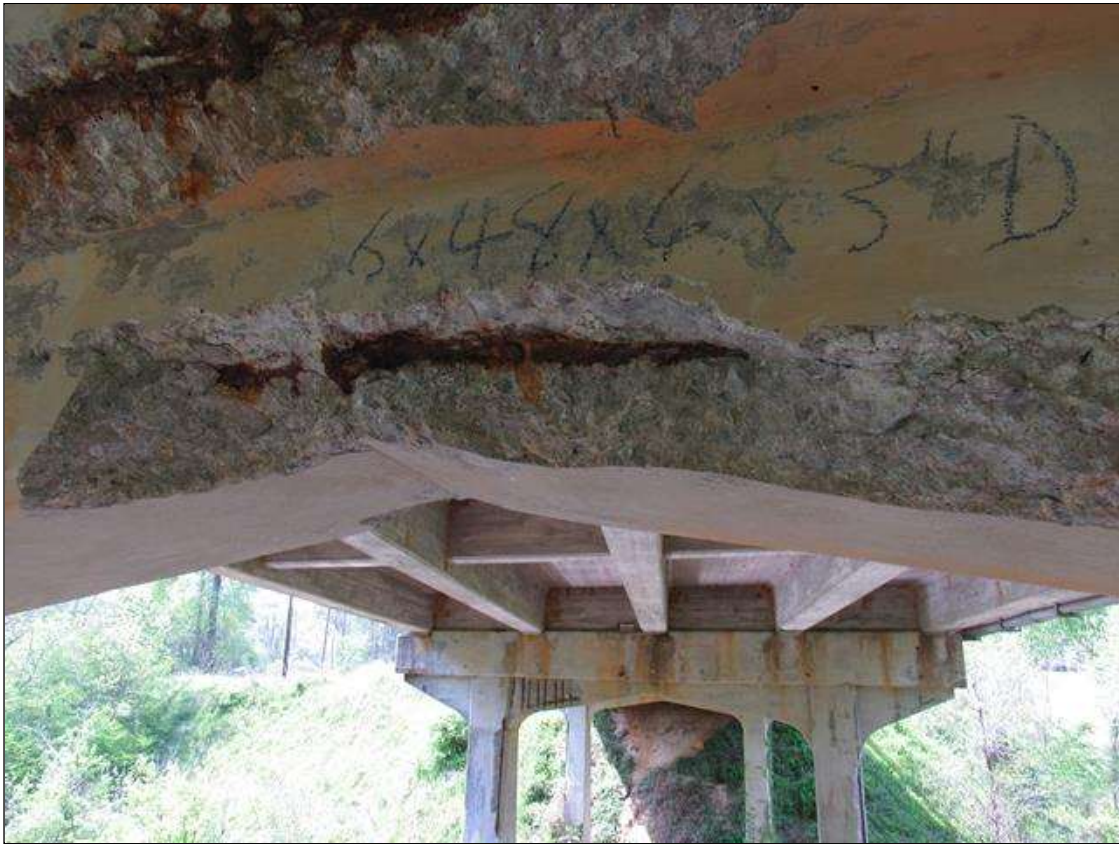
BENT 3 EAST FACE OF HAUNCH UNDER G3 SPALL AND DELAMINATED 6" HIGH 48" LONG 6" UNDER BOTTOM REBAR AND STIRRUPS EXPOSED.
