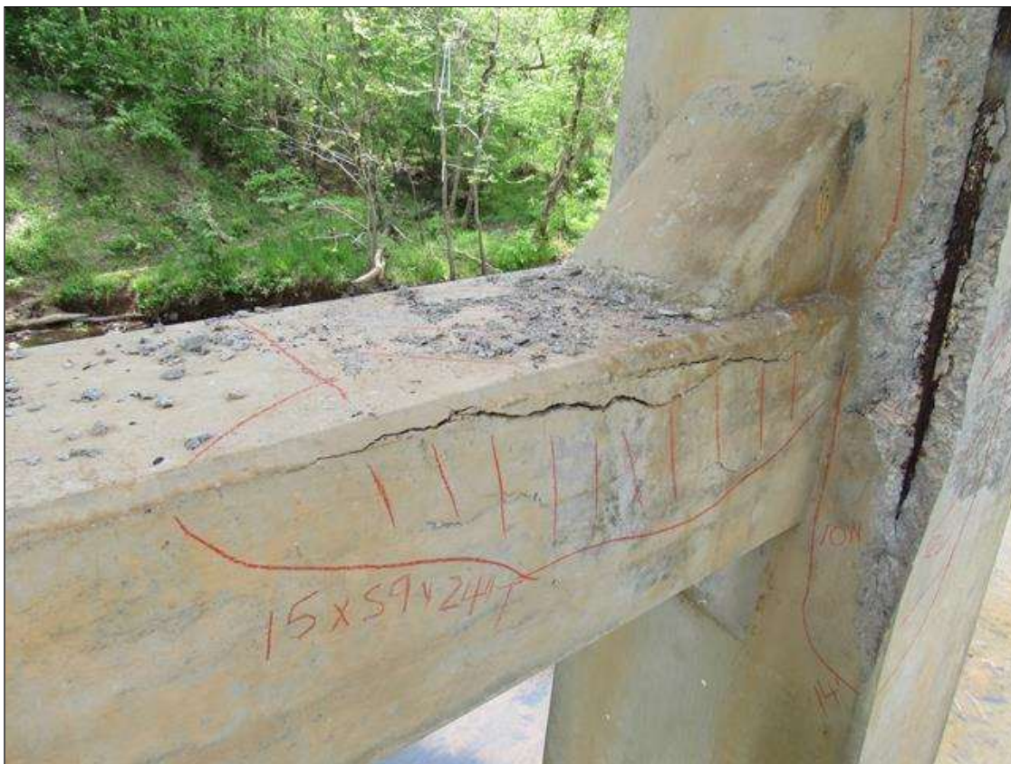
HORZ STRUT BETWEEN PILES 1 AND 2 AT BENT 2 CRACKED AND DELAMINATED AREA LEFT SIDE OF PILE 2 15" DOWN FACE 59" LONG 24" ON TOP.
