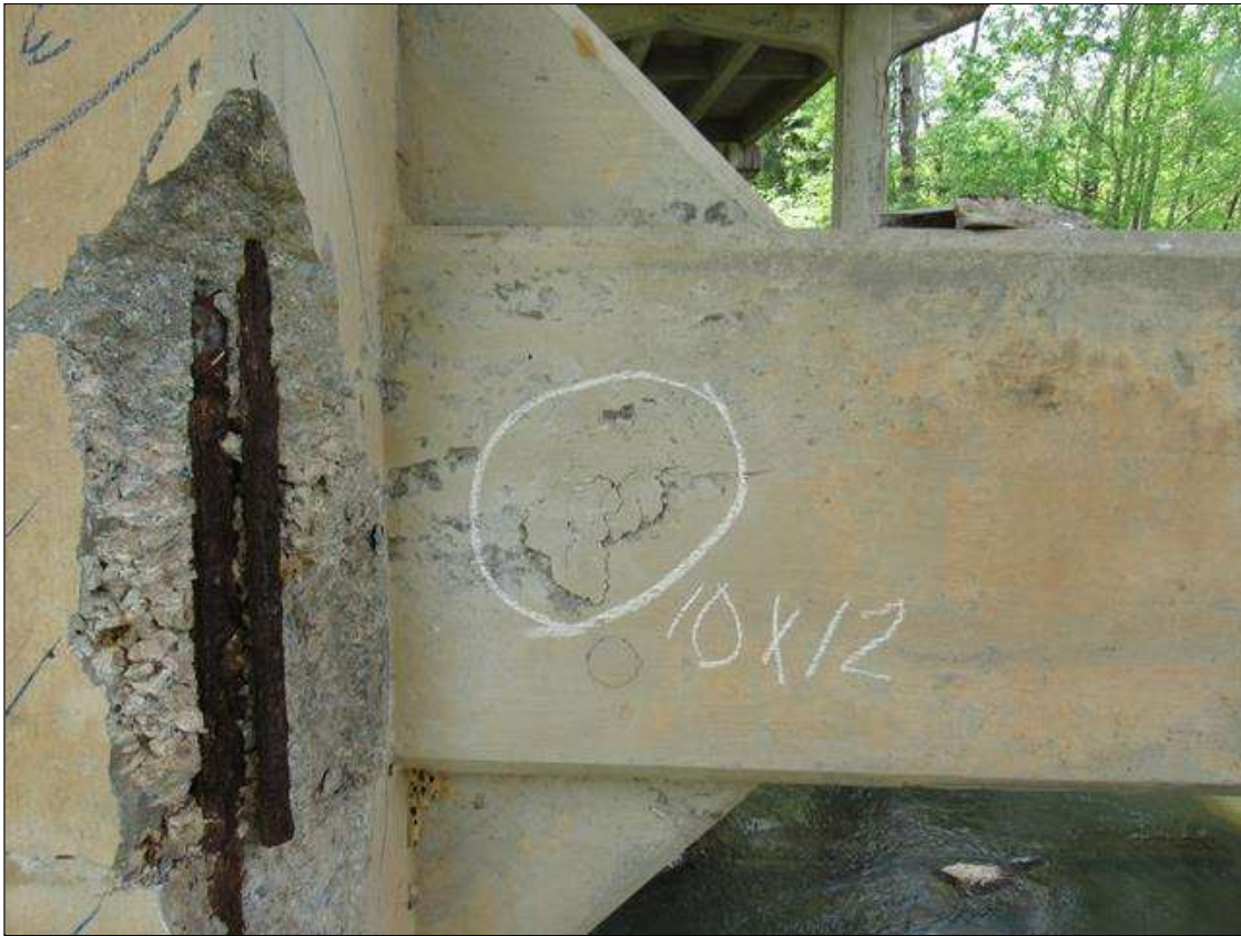
BENT 2 CRACKED DELAMINATED AREA 10" BY 12" ON VERTICAL STRUT RIGHT SIDE OF PILE 1.
