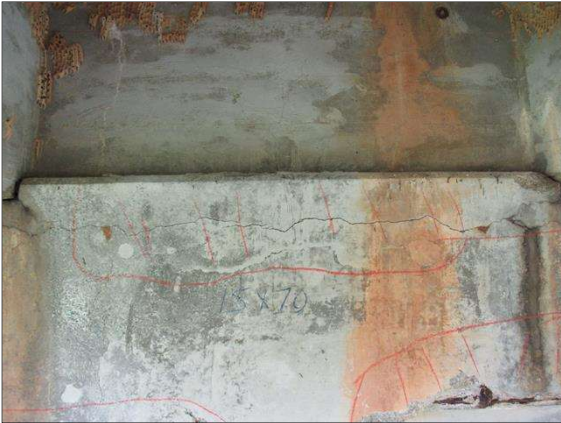
Bent 1 Cap : 6 Feet of Delamination/Spall/Patched Area: Delaminated. Spall 1 inch or less deep or 6 inches or less in diameter. Patched area that is sound BENT 1 WEST FACE OF CAP HAS A HORZ CRACKED DELAMINATED AREA BETWEEN GIRDERS 2 AND 3 ALONG TOP OF CAP. 15" DOWN FACE AND 7" LONG.
