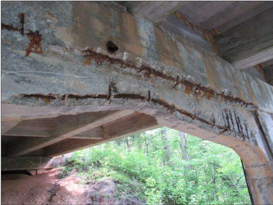
BENT 4 WEST FACE OF HAUNCH CRACKED SPALL DELAMINATED FM 15" TO 24" HIGH 13' 6" LONG 12" UNDER BOTTOM REBAR AND STIRRUPS EXPOSED.
