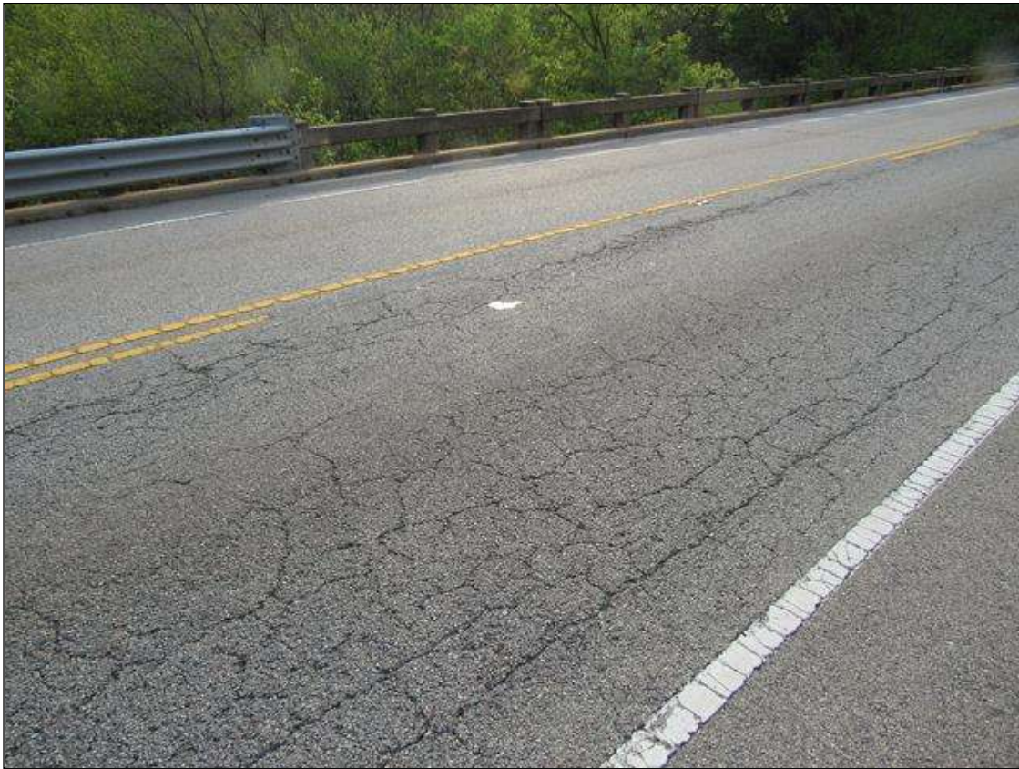
Span 1 Wearing Surface: 1615 Square Feet of Crack (Wearing Surface): Width 0.012-0.05 in. or spacing of 1.0-3.0 ft. SPAN 1 WEARING SURFACE IS HEAVILY MAP CRACKED.
