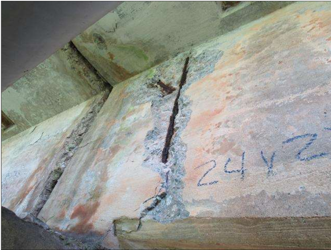
Span 4 Beam 1: 2 Feet of Delamination/Spall/Patched Area: Spall greater than 1 in. deep or greater than 6 in. diameter. Patched area that is unsound or showing distress. Does not warrant structural review. SPAN 4 LEFT SIDE OF G1 OVER BENT 4 CRACKED SPALL DELAMINATED AREA FM END OF GIRDER BACK 24" BOTTOM UP 27" & 1 1/2" DEEP. VERT REBAR EXPOSED.
