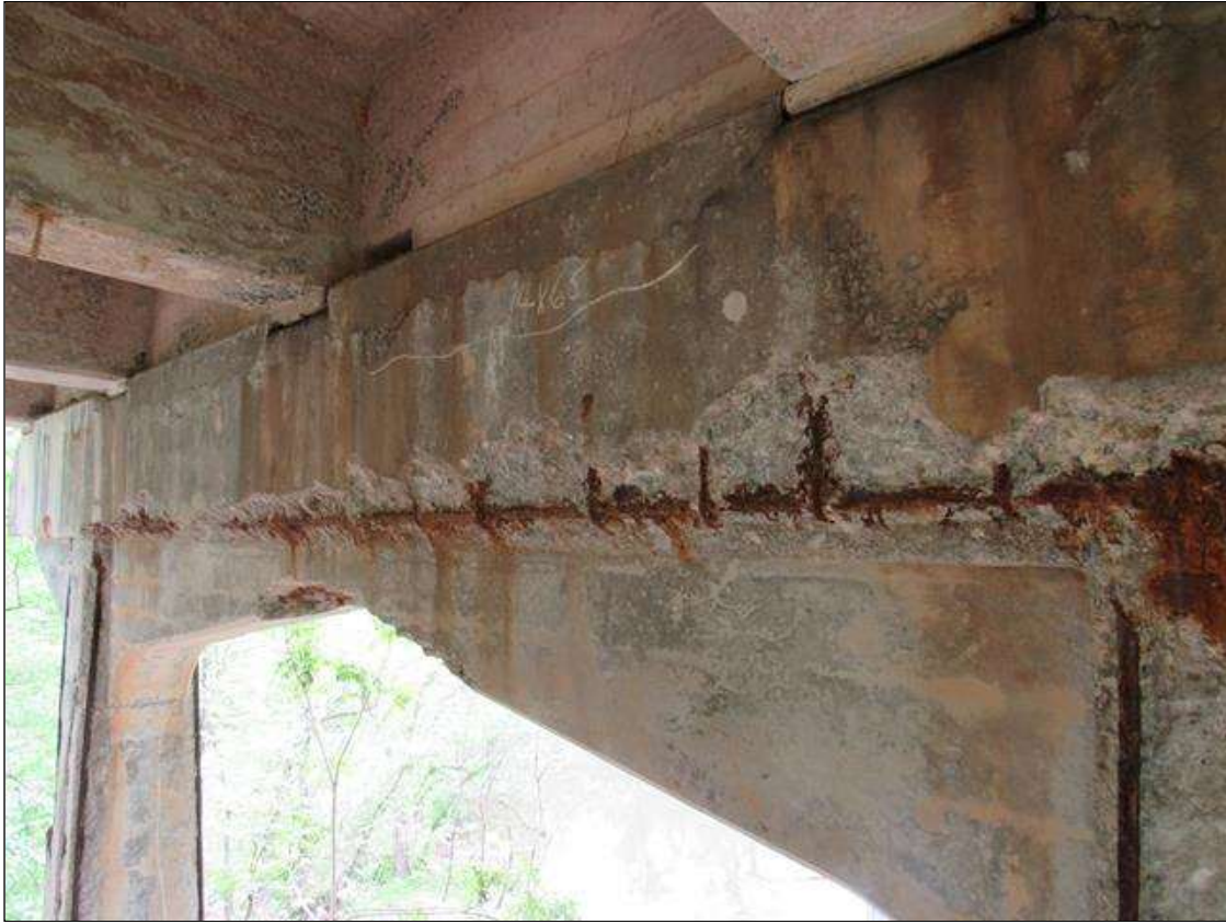
Bent 4 Cap : 0 Feet of Delamination/Spall/Patched Area: Spall greater than 1 inch deep or greater than 6 inches in diameter. PAtched area that is unsound or showing distress. Condition does not warrant structural Review BENT 4 CAP EAST FACE OF CAP CRACKED SPALL DELAMINATED FM LEFT SIDE OF G2 TO RIGHT OF G4. 17" UP FACE 21' LONG 6" UNDER BOTTOM REBAR AND STIRRUPS EXPOSED.
