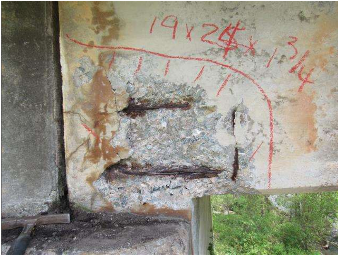
SPAN 2 RIGHT SIDE OF GIRDER 5 HAS A CRACKED SPALL DELAMINATED AREA OVER BENT 1 19" HIGH FM END OUT 24" 1 3/4" DEEP WITH REBAR AND STIRRUPS EXPOSED.
