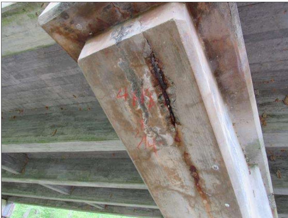
BENT 3 HUANCH AREA UNDER GIRDER 1 HAS A CRACKED AND SPALL AREA WITH REBAR EXPOSED UNDER BOTTOM OF HUANCH. 4" X 18" X 34".
