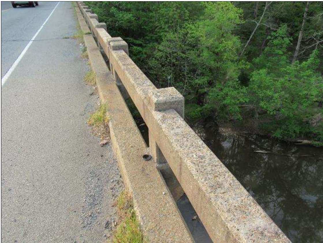
Span 2 Right Bridge Rail: 30 Feet of Cracking (RC and Other): Width 0.012-0.05 in. or spacing of 1.0-3.0 ft. SPAN 2 RIGHT RAIL HAS MAP CRACKING AND SURFACE SCALE TOP OF RAIL AND CURB.
