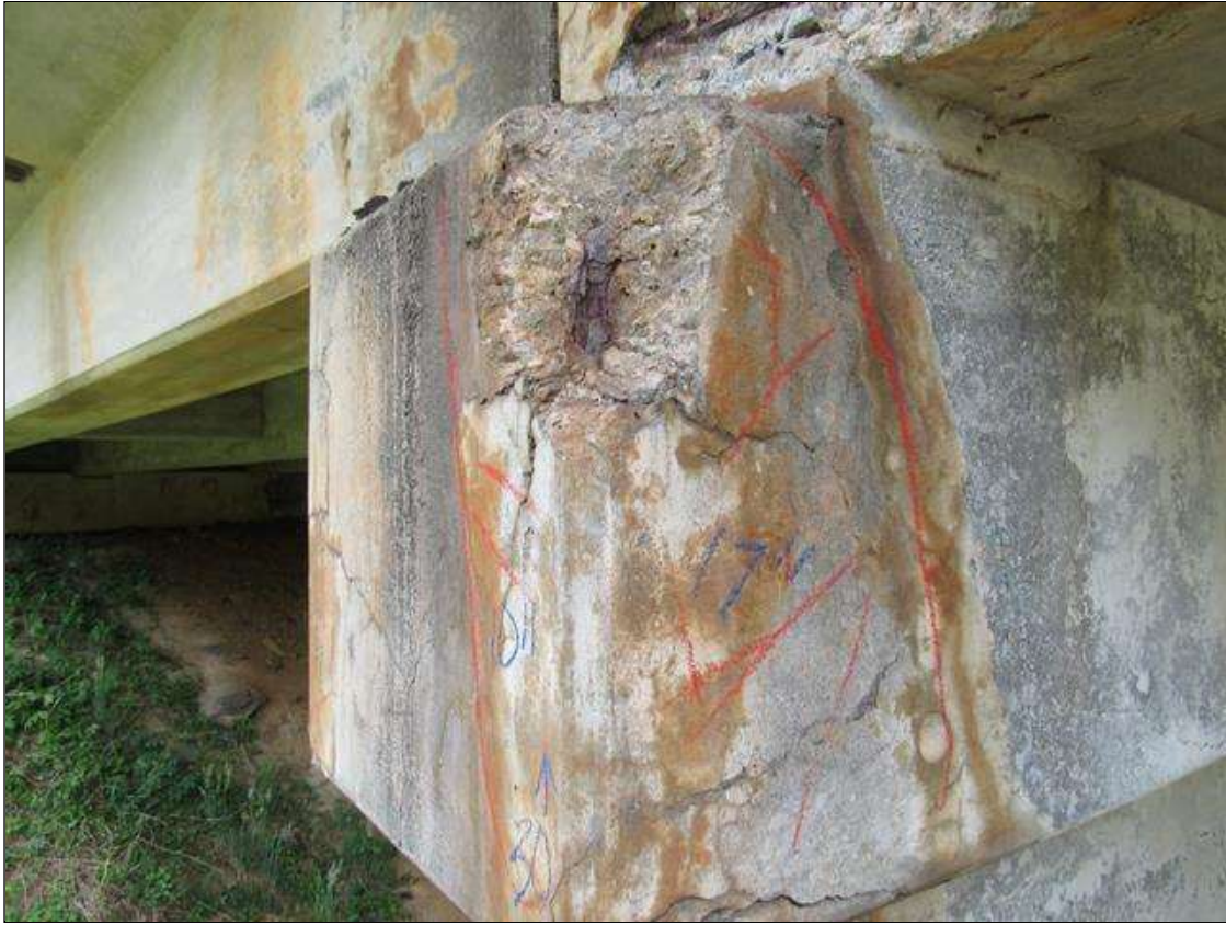
Bent 1 Cap : 0 Feet of Delamination/Spall/Patched Area: Spall greater than 1 inch deep or greater than 6 inches in diameter. Patched area that is unsound or showing distress. Condition does not warrant structural Review BENT 1 RIGHT END AND EAST FACE OF CAP UNDER GIRDER 5 CRACKED SPALL DELAMINATED 10" ON RIGHT END 17" ON EAST FACE TOP DOWN 30".
