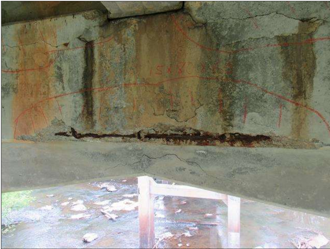
Bent 1 Cap : 7 Feet of Delamination/Spall/Patched Area: Delaminated. Spall 1 inch or less deep or 6 inches or less in diameter. Patched area that is sound BENT 1 WEST FACE OF CAP HAS A HAS CRACKED DELAMINATED SPALL AREA UNDER G3 15" UP BASE 80" LONG AND 6" UNDER BOTTOM. LARGE REBAR AND STIRRUPS EXPOSED.
