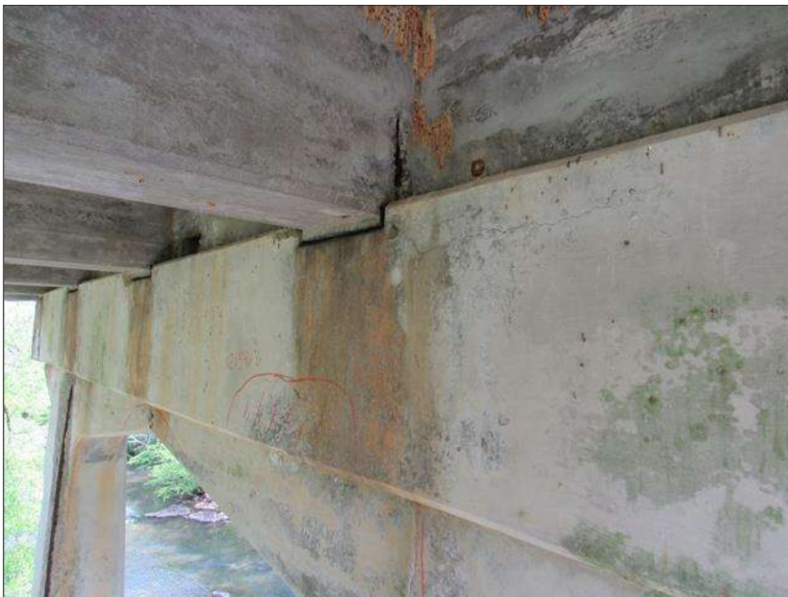
Bent 2 Cap : 15 Feet of Delamination/Spall/Patched Area: Delaminated. Spall 1 inch or less deep or 6 inches or less in diameter. Patched area that is sound BENT 2 WEST FACE OF CAP HAS HORZ CRACKS ALONG THE TOP AND MAP CRACKING ON THE ENDS.
