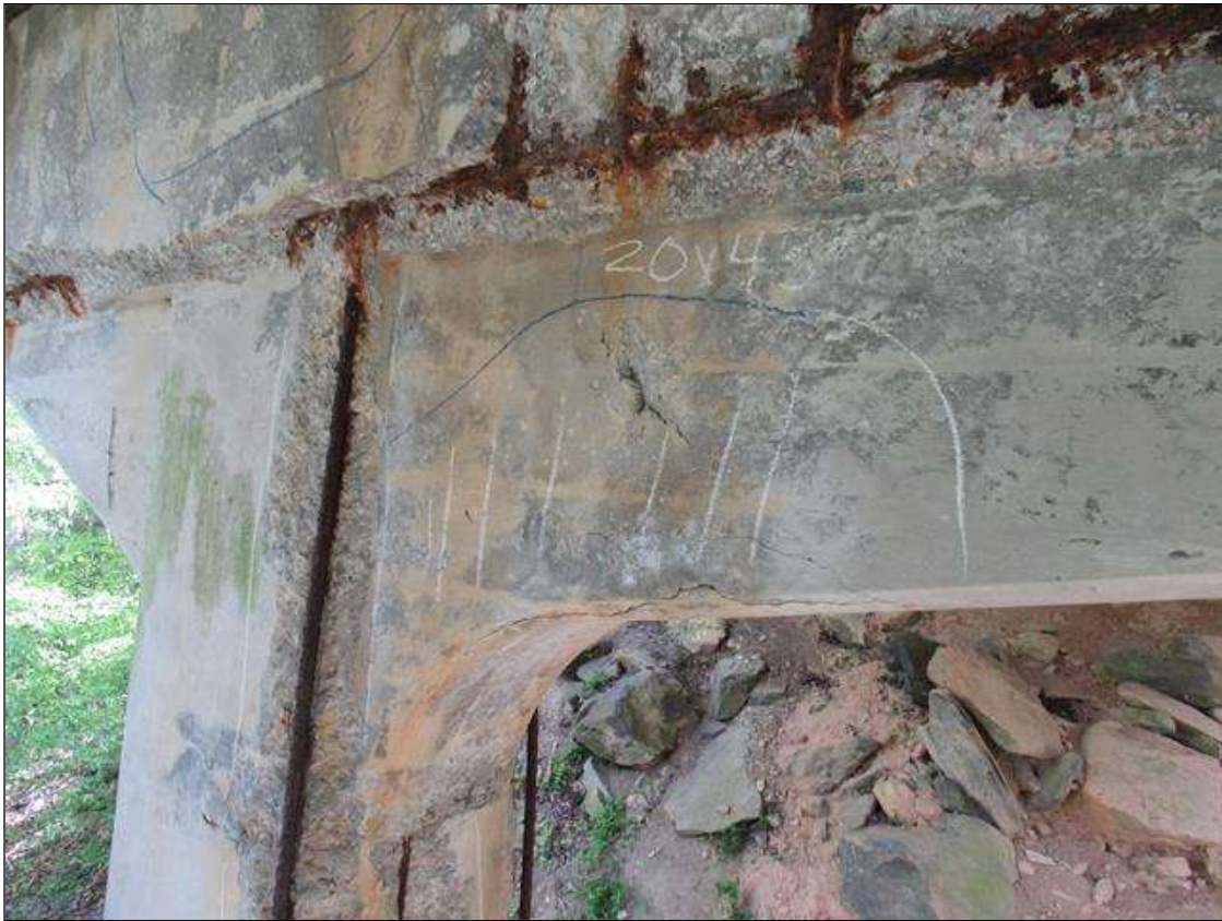
BENT 4 WEST FACE OF HAUNCH RIGHT SIDE OF PILE 1 CRACKED DELAMINATED 20" X 43" AND 10" UNDER BOTTOM.
