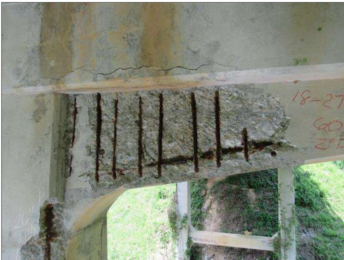
BENT 2 EAST FACE OF HAUNCH UNDER BOTTOM OF CAP LEFT OF PILE 2 CRACKED SPALL AND DELAMINATED. 18" TO 27" DOWN FACE 60" LONG 2" DEEP WITH STIRRUPS AND REBAR EXPOSED.
