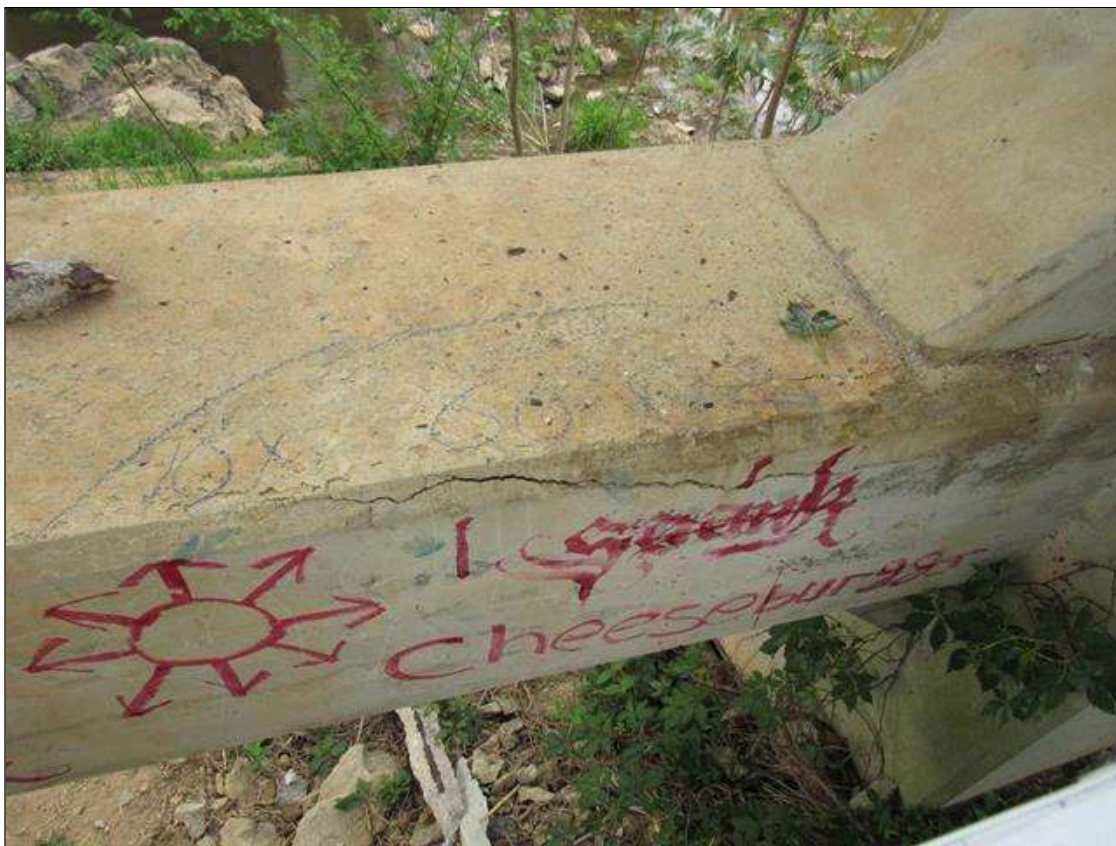
HORZ STRUT BEWTEEN PILE 1 AND 2 HAS A CRACKED AND DELAMINATED AREA ON TOP AND WEST FACE LEFT SIDE OF PILE 2 10" ON TOP 60" LONG AND 12" ON WEST FACE.
