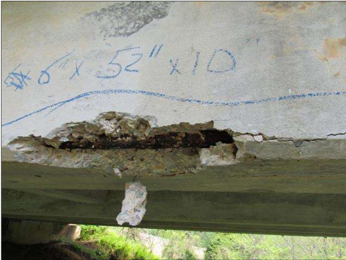
SPAN 1 GIRDER 5 HAS A CRACKED SPALL DELAMINATED AREA LOCATED AT 15' FM BENT 1. 6" UP FACE 52" LONG 10" UNDER BOTTOM WITH LARGE REBAR EXPOSED.
