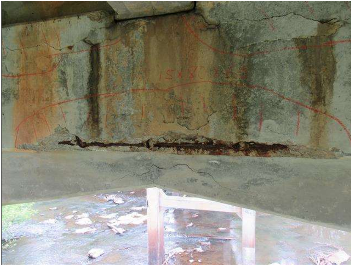
BENT 1 WEST FACE OF CAP HAS A HAS CRACKED DELAMINATED SPALL AREA UNDER G3 15" UP BASE 80" LONG AND 6" UNDER BOTTOM. LARGE REBAR AND STIRRUPS EXPOSE
