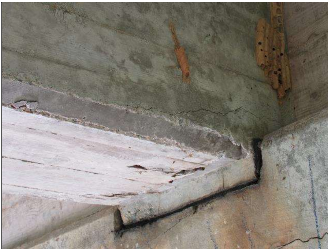
Span 4 Beam 4: 2 Feet of Cracking (RC and Other): Width 0.012-0.05 in. or spacing of 1.0-3.0 ft. SPAN 4 LEFT SIDE OF G4 AT BENT 3 CRACKED AND DELAMINATED AREA ALONG BOTTOM OF GIRDER. 3" UP FACE FROM END OF GIRDER OUT 17" AND 2" UNDER BOTTOM.
