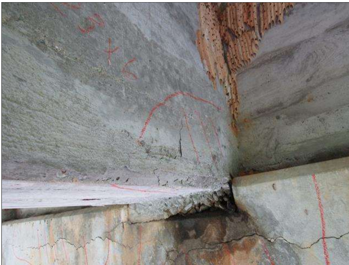
Span 3 Beam 3: 2 Feet of Delamination/Spall/Patched Area: Delaminated. Spall 1 in. or less deep or 6 in. or less in diameter. Patched area that is sound. SPAN 3 GIRDER 3 LEFT SIDE HAS CRACKED DELAMINATED AREA FM BENT 2 CAP OUT 23".
