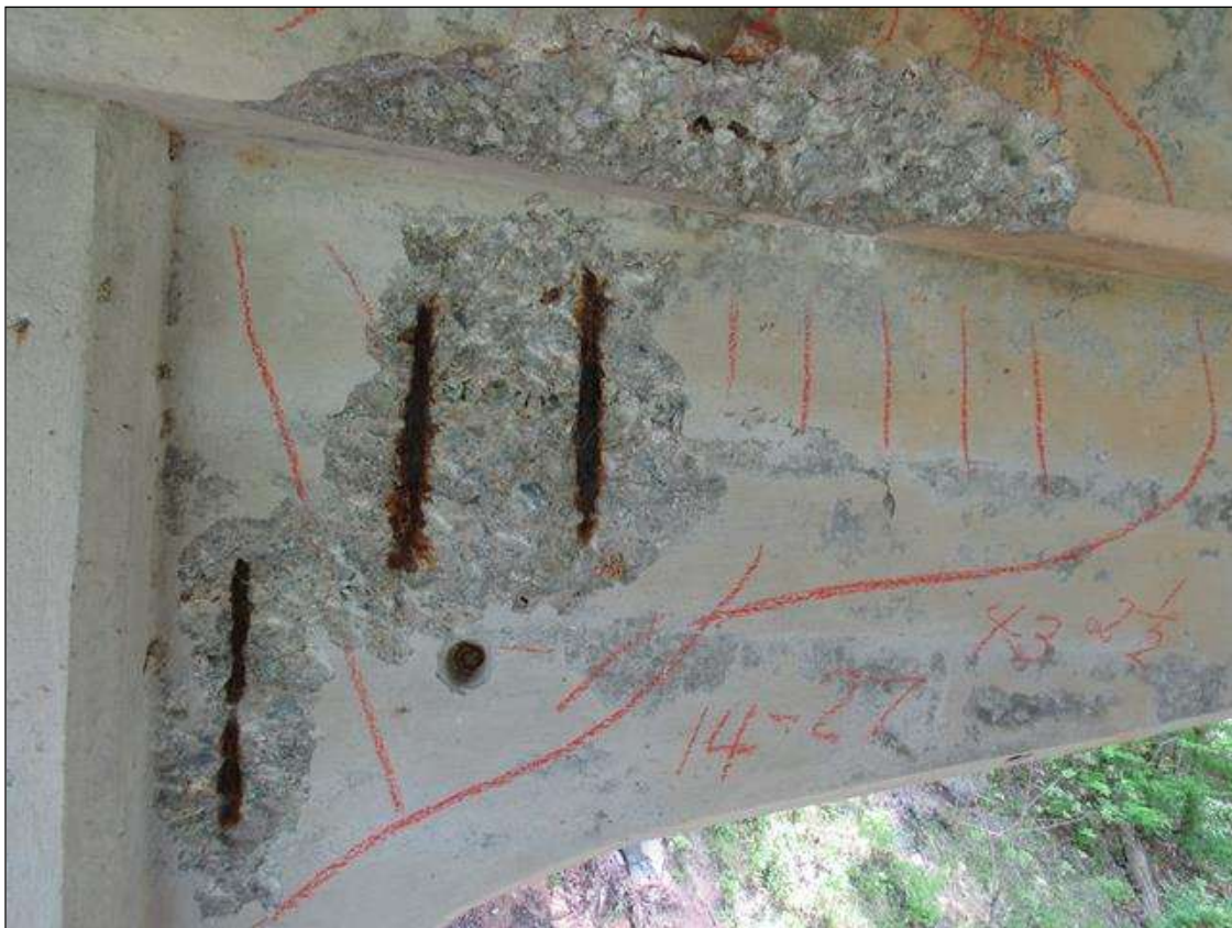
BENT 3 WEST FACE OF HAUNCH RIGHT SIDE OF PILE 1 CRACKED SPALL DELAMINATED. 14" TO 27" DOWN FACE 43" LONG 2 1/2" DEEP REBAR EXPOSED.
