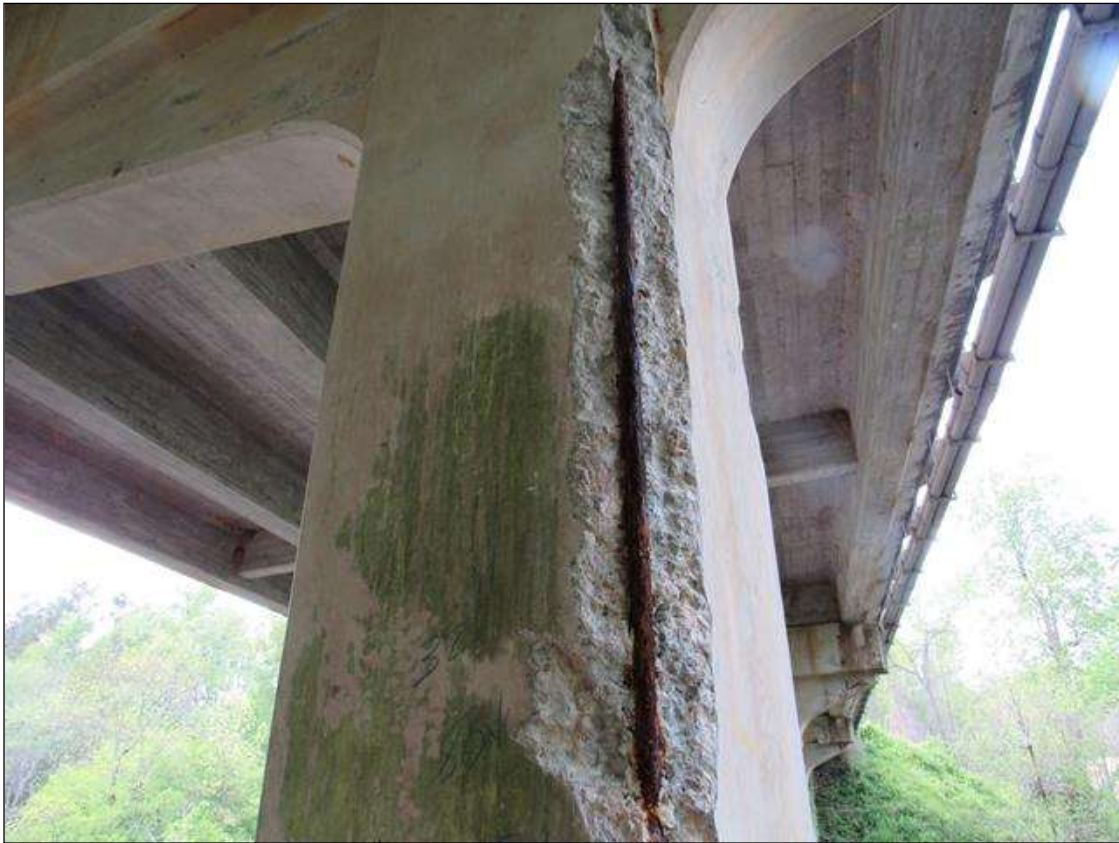
BENT 3 PILE 1 CRACKED SPALL DELAMINATED AREA NE CORNER OF PILE STARTS 32" BELOW CAP EXTENDS DOWN 80" 11" ON EAST AND 6" NORTH.
