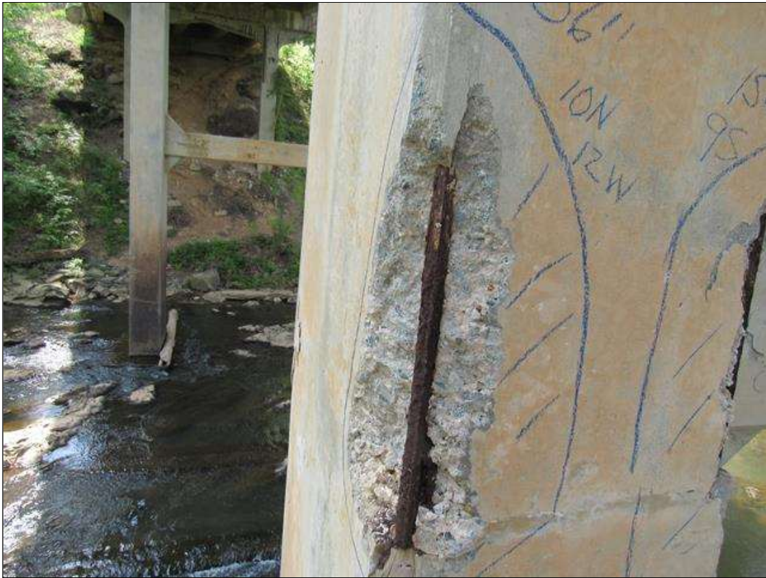
Bent 2 Pile 1: 0 Each of Delamination/Spall/Patched Area: Spall greater than 1 in. deep or greater than 6 in. diameter. Patched area that is unsound or showing distress. Does not warrant structural review. BENT 2 PILE 1 NW CORNER HAS CRACKED SPALL DELAMINATED AREA START 15' ABOVE FOOTING EXTENDS UP 36" & 10" ON NORTH FACE 12" ON WEST FACE WITH 2 LARGE REBAR EXPOSED.
