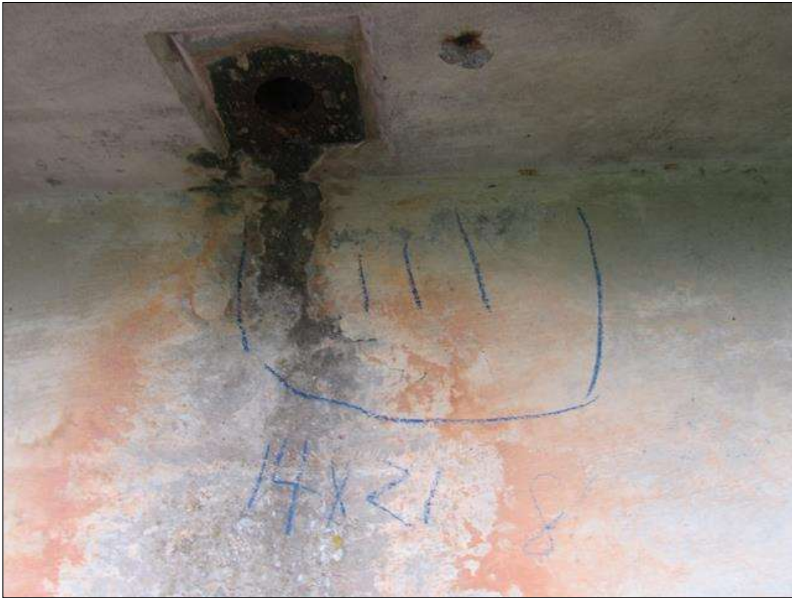
Span 4 Beam 5: 2 Feet of Delamination/Spall/Patched Area: Delaminated. Spall 1 in. or less deep or 6 in. or less in diameter. Patched area that is sound. SPAN 4 RIGHT SIDE OF G5 HAS A CRACKED DELAMINATED AREA IN FACE OF GIRDER 8' FROM BENT 4 CAP 14" X 21".
