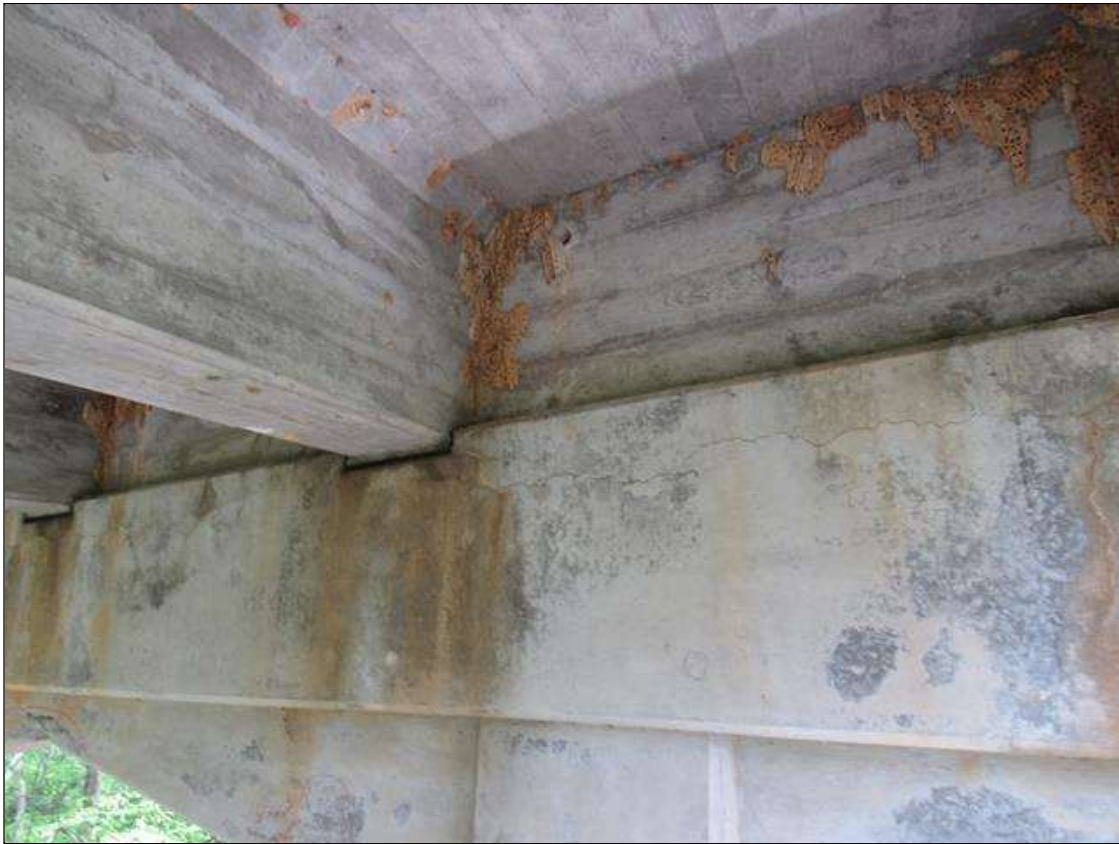
Bent 3 Cap : 24 Feet of Cracking (RC and Other): Width 0.012-0.05 in. or spacing of 1.0-3.0 ft. BENT 3 CAP WEST FACE HAS HORZ CRACKS ALONG TOP EDGE FROM G1 TO G5 AND APPROX 10" TO 12" DOWN FACE.
