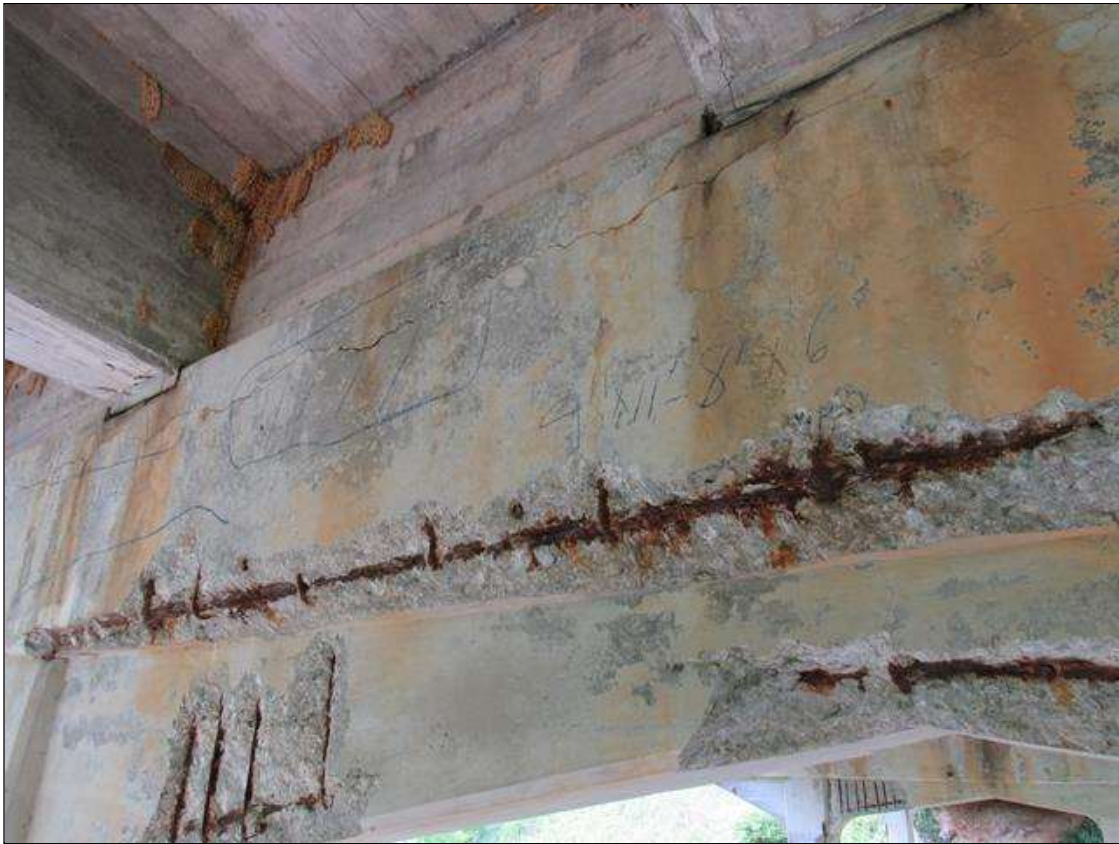
Bent 3 Cap : 0 Feet of Delamination/Spall/Patched Area: Spall greater than 1 inch deep or greater than 6 inches in diameter. Patched area that is unsound or showing distress. Condition does not warrant structural Review BENT 3 EAST FACE OF CAP HAS A DELAMINATED AND SPALL AREA ALONG BOTTOM EDGE OF CAP FM G3 TO RT OF G4. 9" UP FACE 11' 8" LONG 6" UNDER BOTTOM REBAR STIRRUPS EXPOSED.
