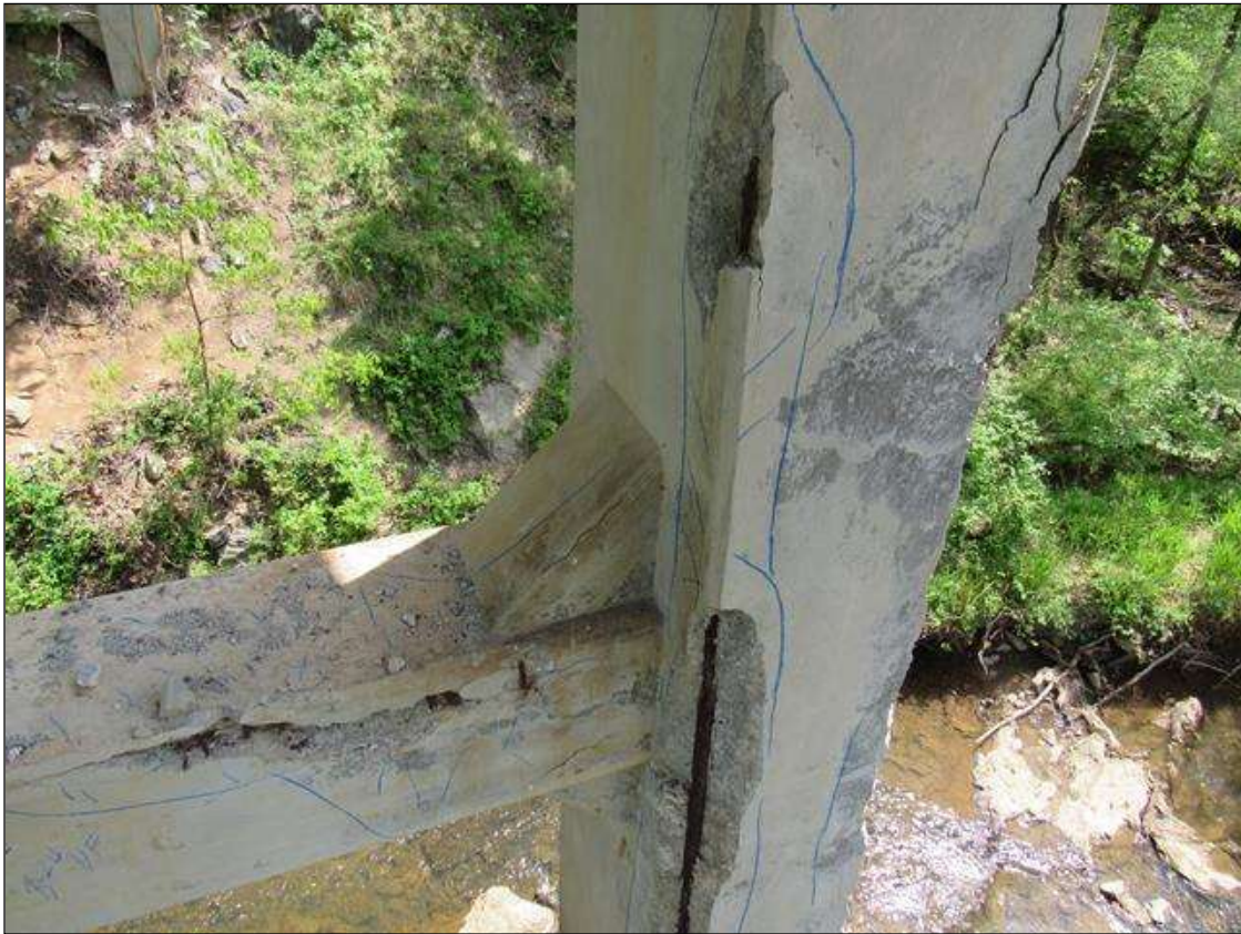
BENT 3 PILE 2 CRACKED SPALL DELAMINATED AREA NW CORNER STARTS 12' ABOVE FOOTING EXTENDS UP 11' 6". 16" ON NORTH AND 11" ON WEST.
