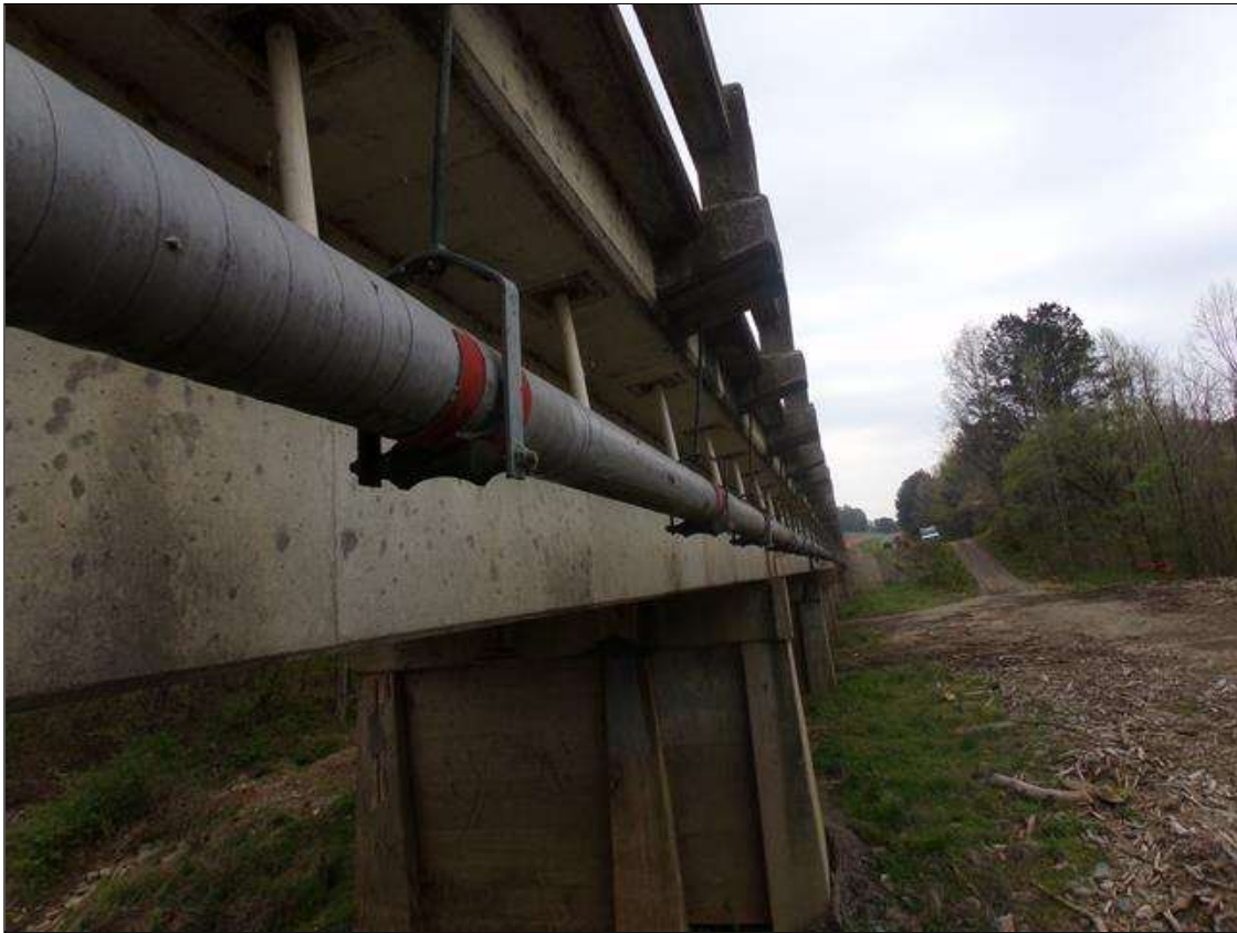
Utility under west overhang
