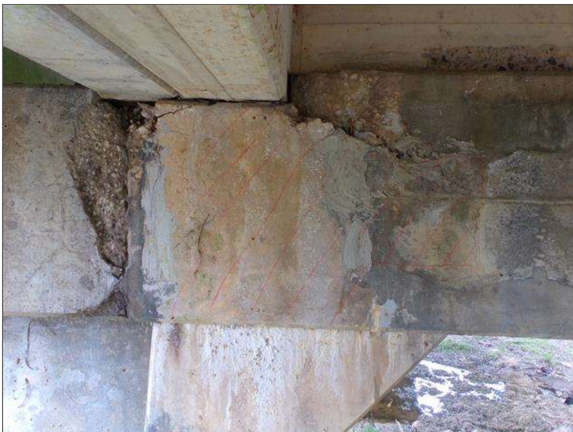
Bent 3 Cap 1: 6' long x up to full height area of delamination on south face of cap under beam 3 in to bay 2.
