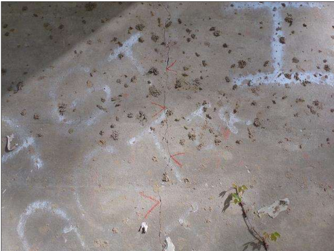
Full height vertical crack in web wall up to 1/8" wide between columns 2 and 3 south face.
