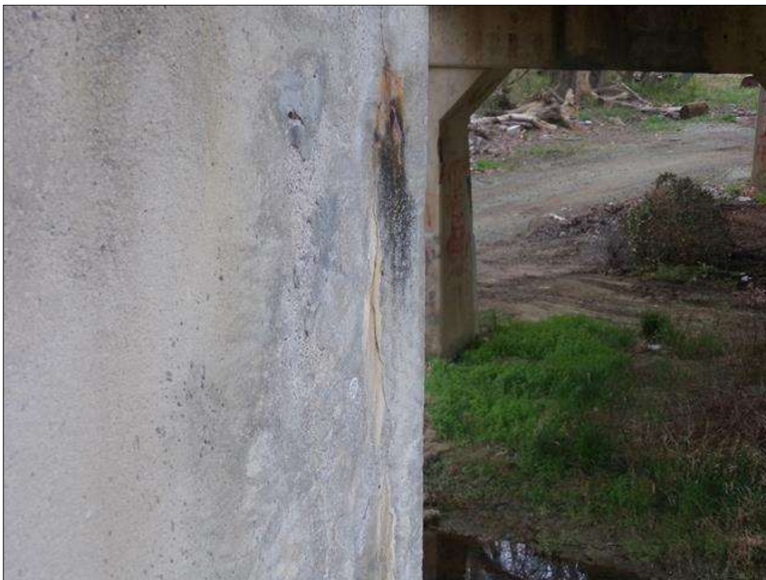
Bent 4 Cap 1: Full height vertical crack up to 1/16" wide on west face of cap.
