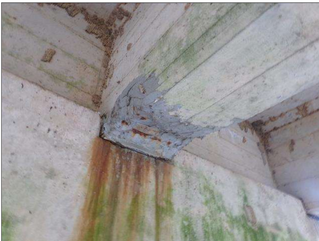
Span 5 Beam 4: 1' long x full width of bottom of beam sound patched area with staining at pier 5.
