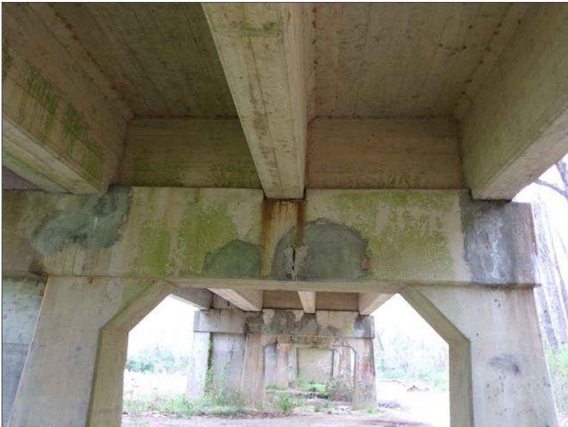
Bent 1 Cap 1: Several sound patched area on south face of cap up to 4' square starting under beam 2.
