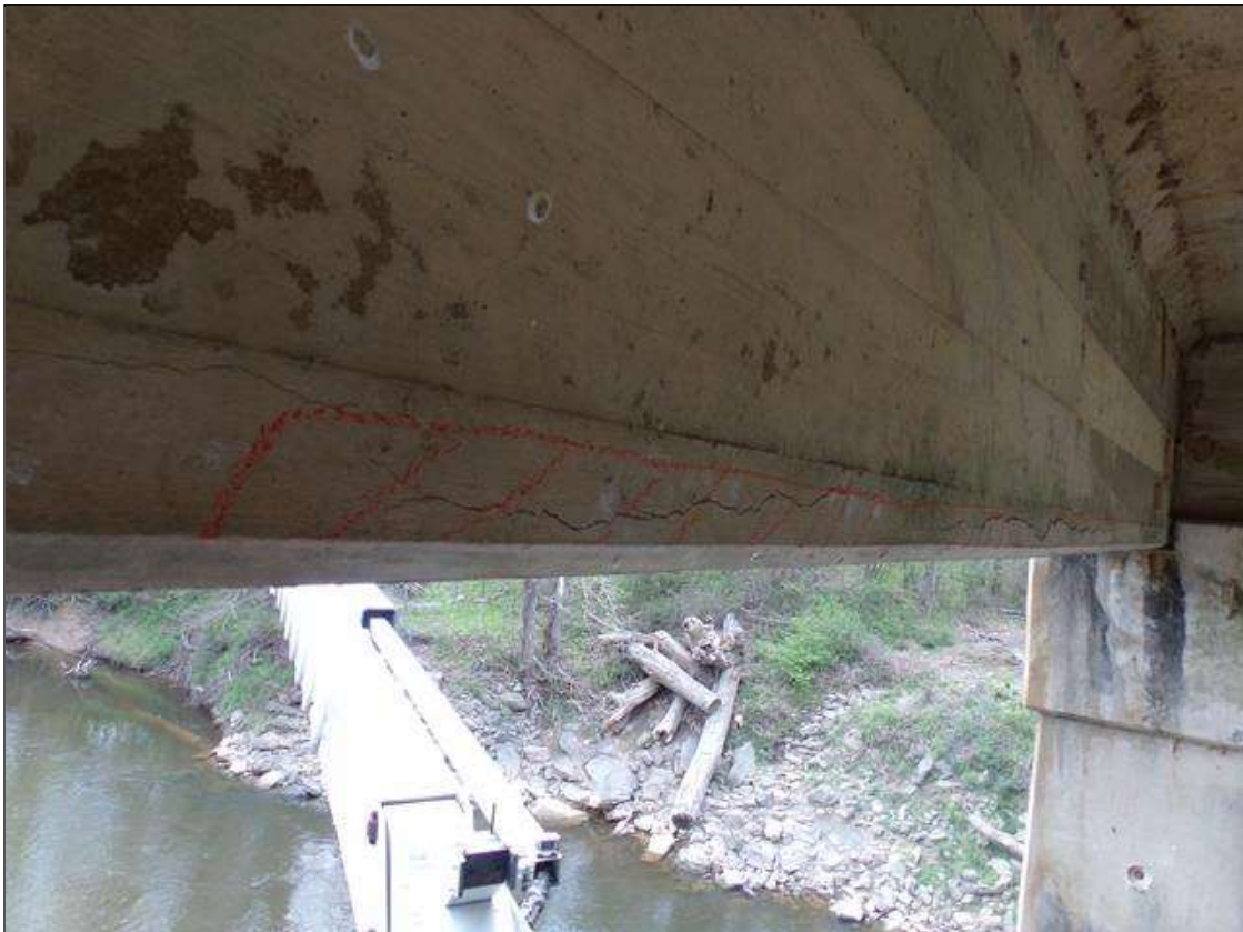
Span 6 Beam 5: 10' long x 4" high area of delamination with a full length cracks up to 1/4" wide on west face of bottom of beam starting 10' from pier 5.
