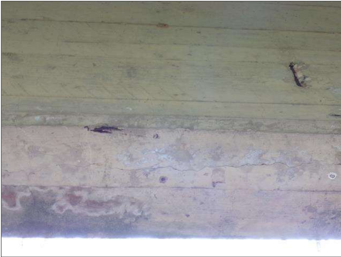
Span 1 Beam 5: 3' long longitudinal crack up to 1/16" wide on bottom of beam at mid span.
