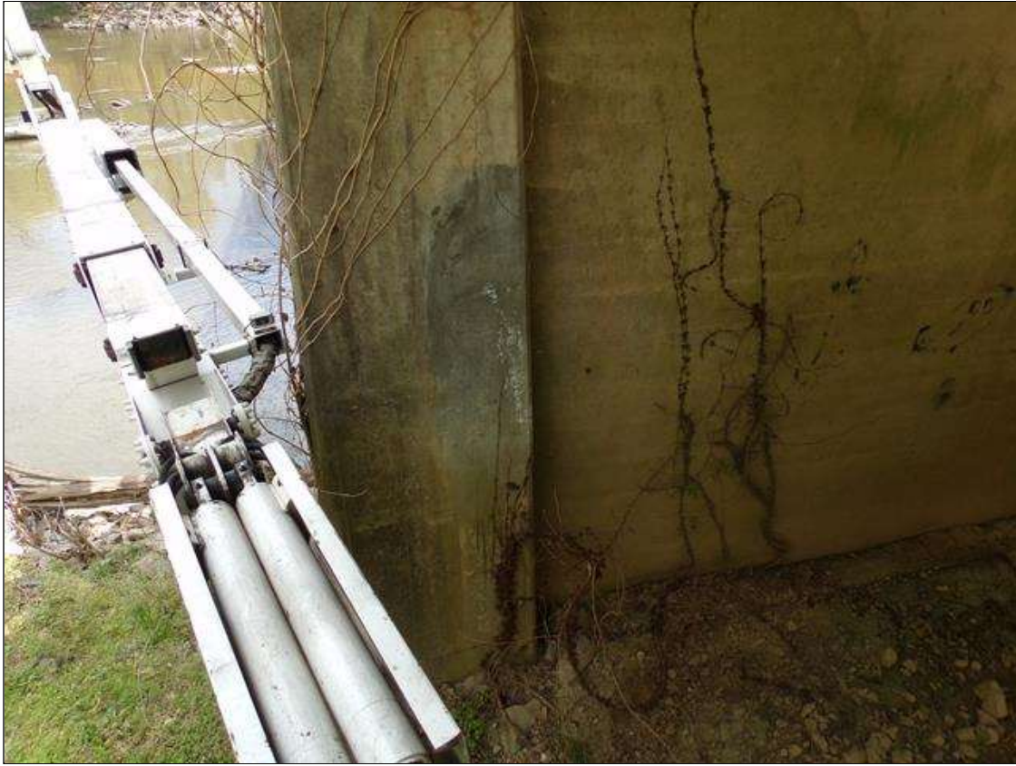
Bent 9 Pile 3: 5' high x 1' wide sound patched area on north face of column starting 3' from ground line.
