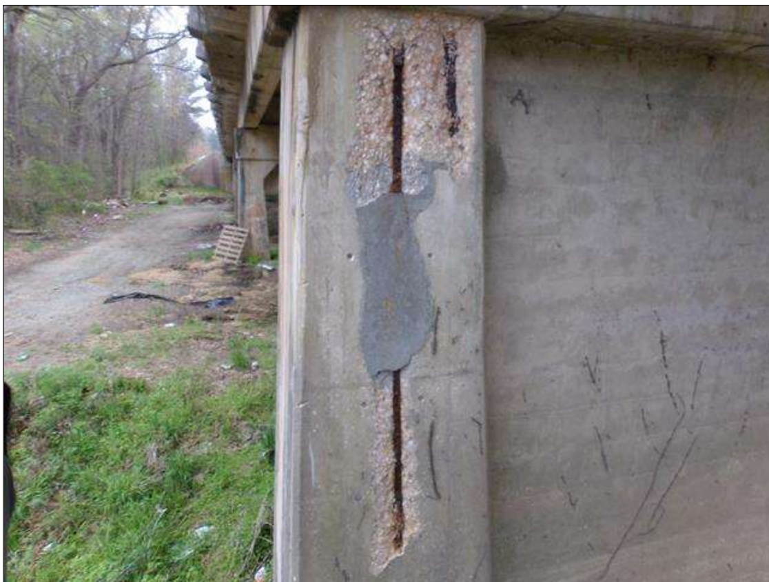
Bent 4 Pile 1: PM-- Patch that has failed, Spall 8' long x up to 21" wide x 2" deep with exposed rebar with section loss on north face of column starting under cap.
