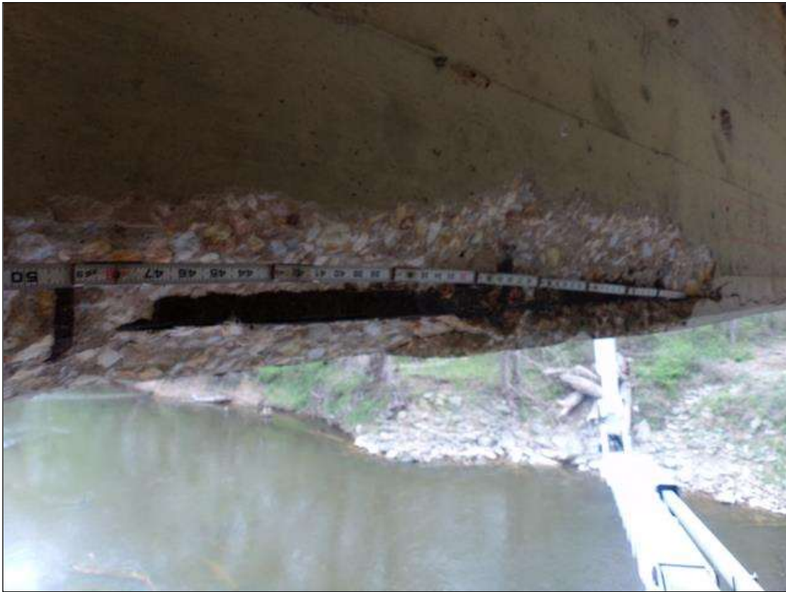
Span 6 Beam 5: PM--Spall 4' long x 10" high on west face x 8" wide on bottom of beam with exposed rebar with section loss 14' from pier 6.
