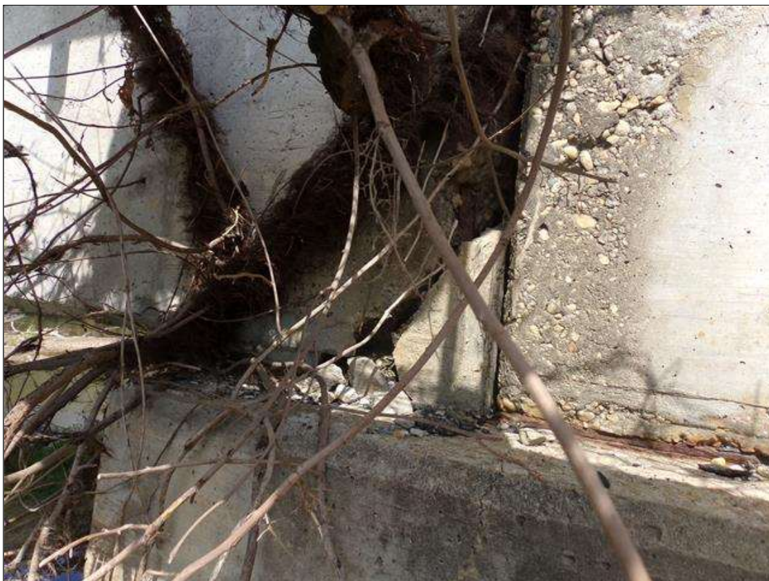
Span 4 Beam 1: 1' high x 7" wide x full width bottom corner spall at end of beam with exposed rebar with no measurable section loss over pier 3.
