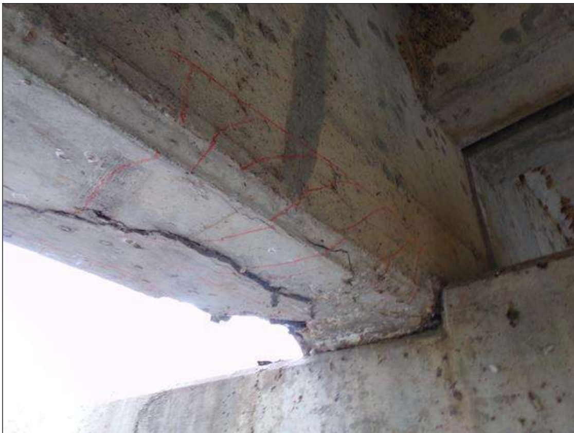
Span 5 Beam 1: 2' long x 14" wide on bottom of beam x 6" high on east face area of delamination starting at pier 5
