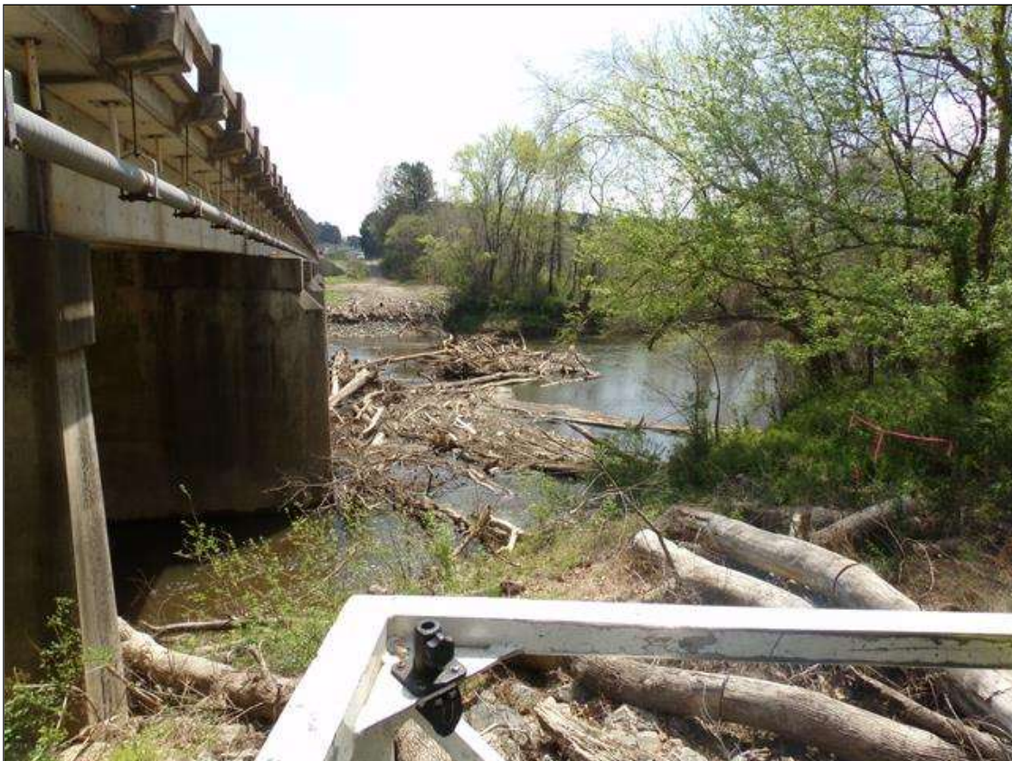
Drift accumulation at upstream end of bridge 200' long x 100' wide x 8' high, removal process has been started.
