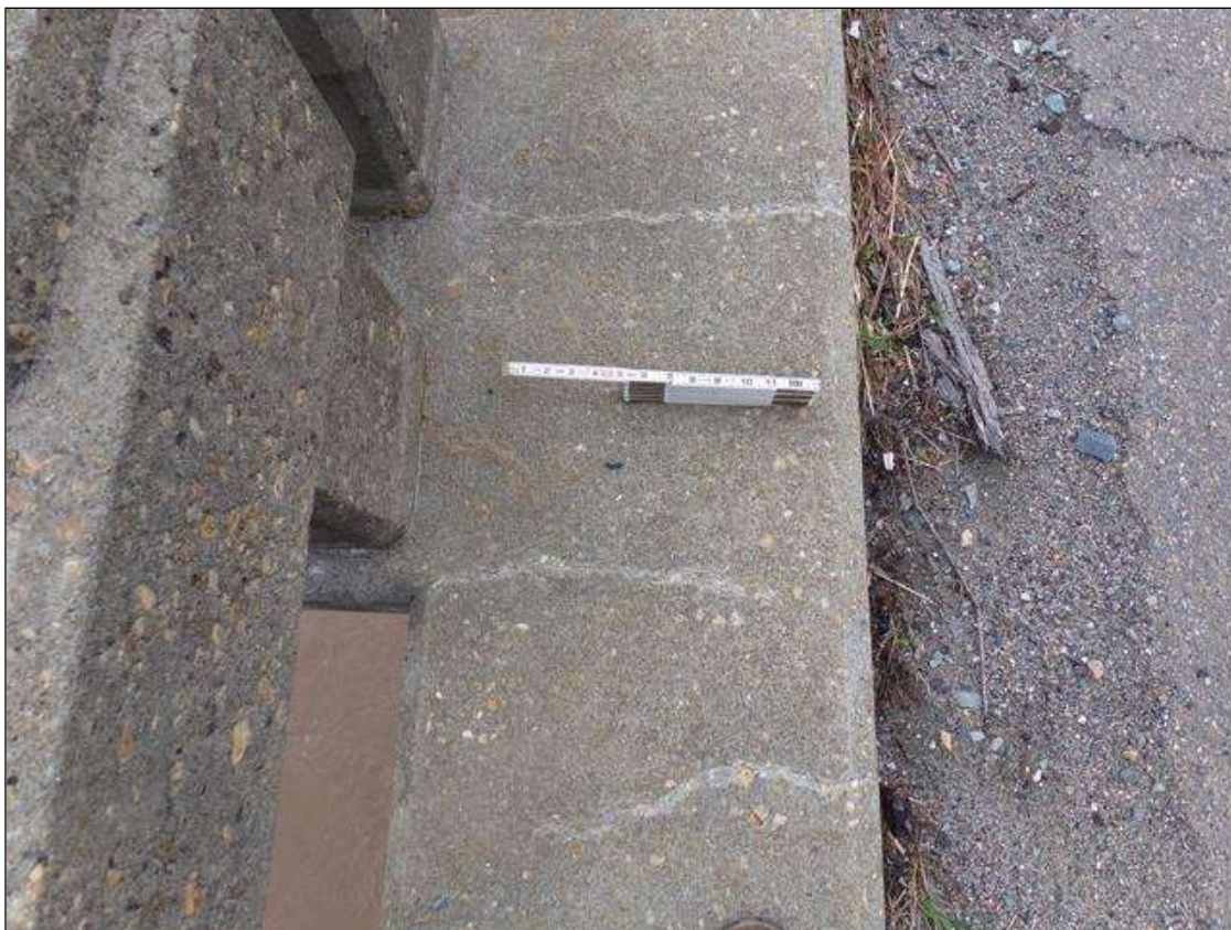
Typical full/partial width transverse cracks in top of curb at various locations right rail only all spans, span 8 shown.
