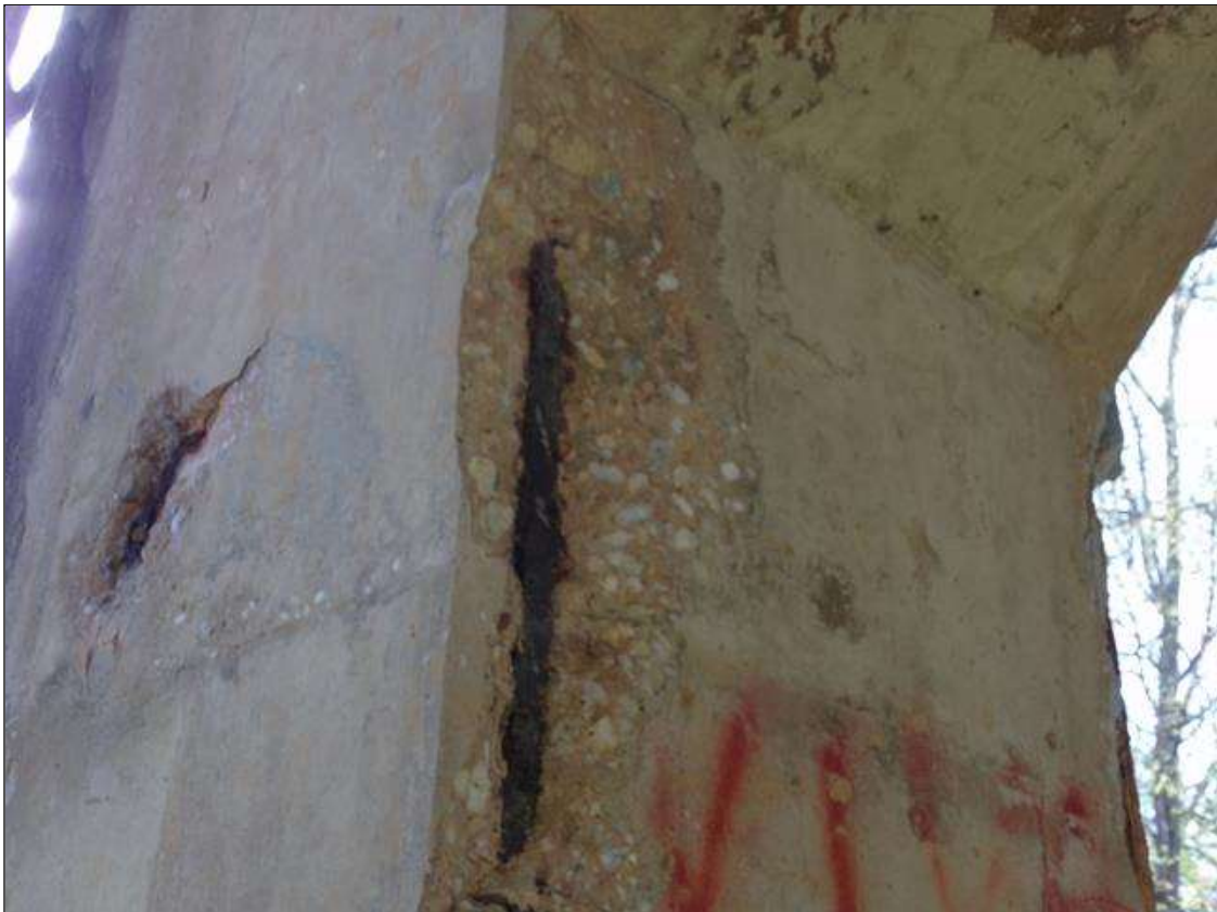
Bent 3 Pile 3: 27" high x 9" wide x 1 1/2" deep spall with exposed rebar with no measurable section loss on west face of column starting 6' from ground.
