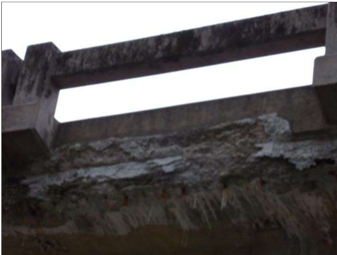
Span 2 Right Bridge Rail: East face of curb has several failed patched areas that have spalled out up to 5' long x 8" high x 2" deep at various locations.
