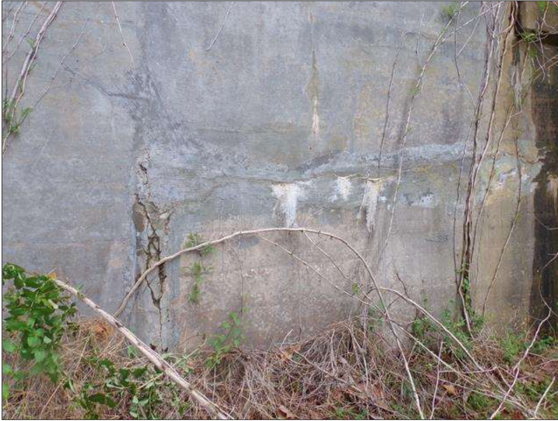
End Bent 2 Abutment/Backwall : Patched area 24' long x up to 6' high starting 12' from west end that is unsound with full width horizontal crack up to 3/16" wide with efflorescence and an area of map cracking at west end of patch up to 1/8" wide.
