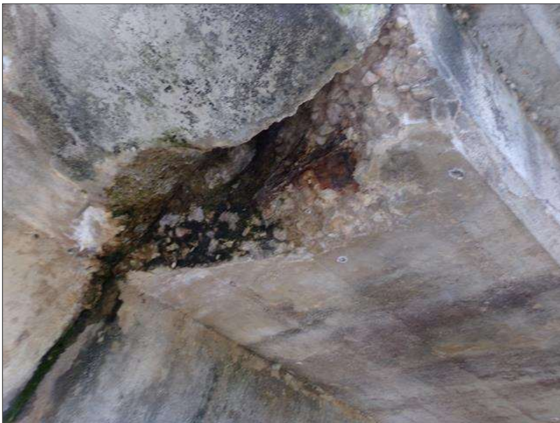
Span 9 Deck: Spall in east overhang 2' wide x 9" long x 5" deep with exposed rebar with no measurable section loss at end of span over pier 8.
