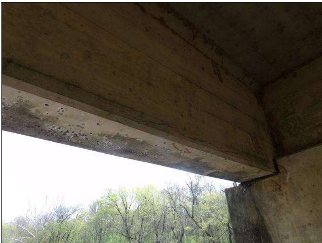
Span 8 Beam 5: Delamination 4' long x up to full width of bottom of beam x 4" high on west face starting 1' from pier 7
