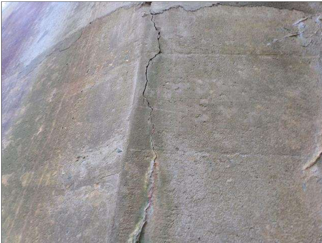
End Bent 1 Abutment/Backwall : Full height vertical/diagonal crack up to 1/16" wide with efflorescence starting at top of abutment 4' from beam 5 east side.
