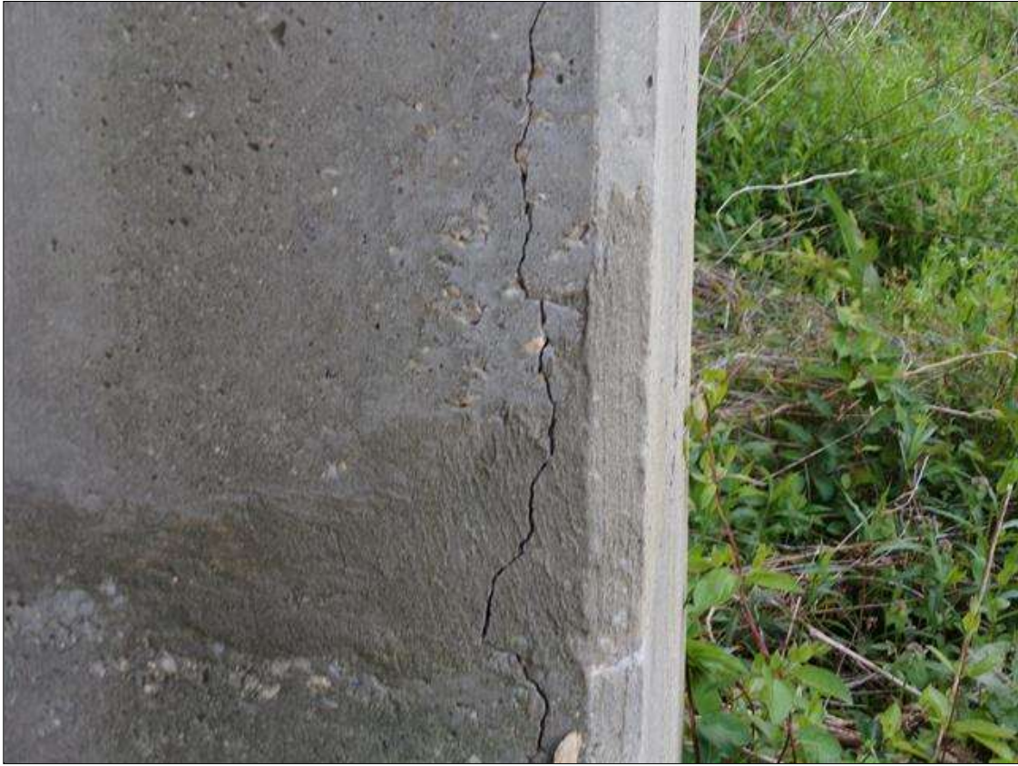
Bent 1 Pile 1: 3' high vertical crack up to 1/8" wide on north face of column starting 2' from ground line.
