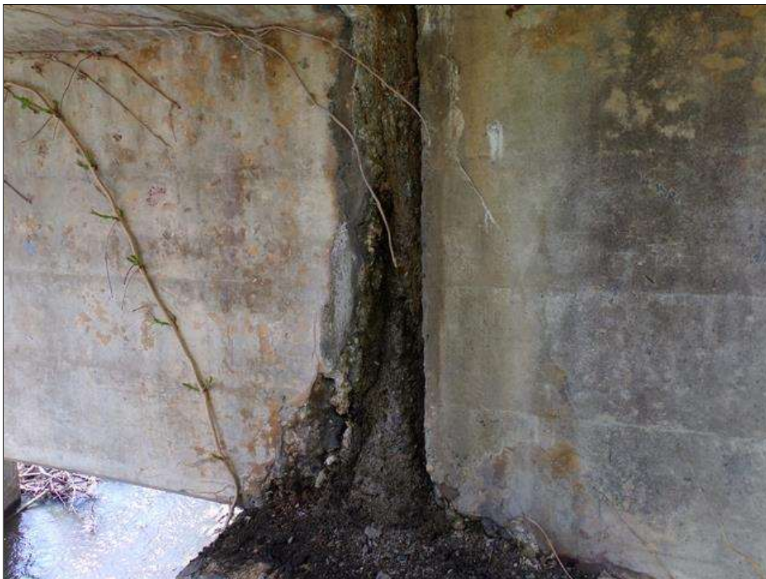
Span 9 Beam 5: Up to 1' long x full height at end of beam area of concrete deterioration with spalling up to 3" deep starting at pier 9.
