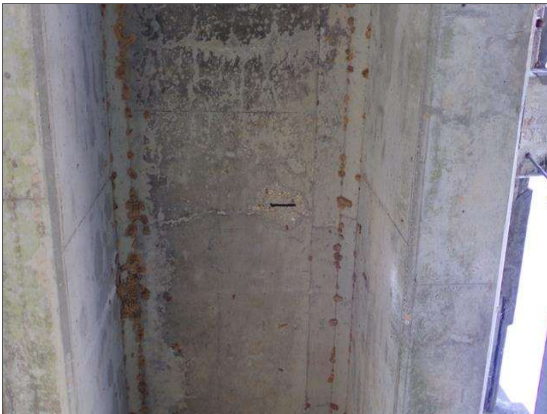
Span 3 Deck: 1' diameter spall 3/4" deep with exposed rebar with no measurable section loss on underside of deck in bay 1, 16' from middle diaphragm
