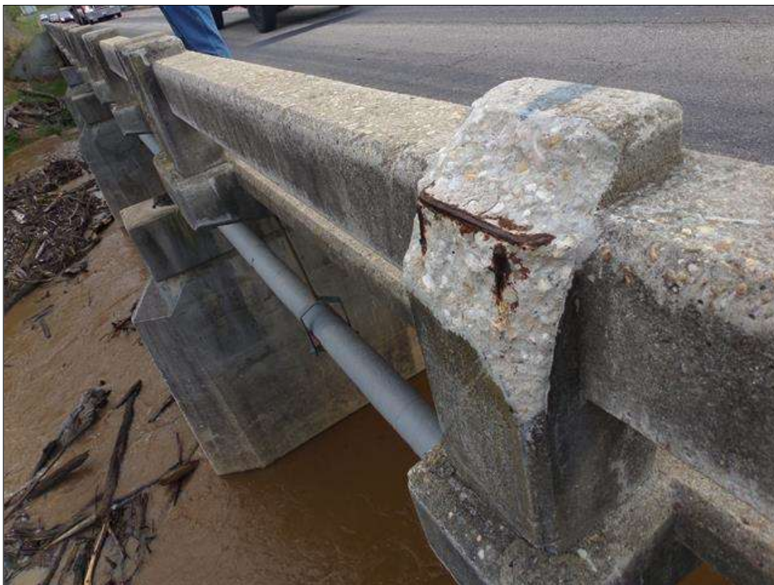
Span 6 Left Bridge Rail: 1' high x full width x 2" deep spall with exposed rebar with no measurable section loss in top of rail post 5 west face
