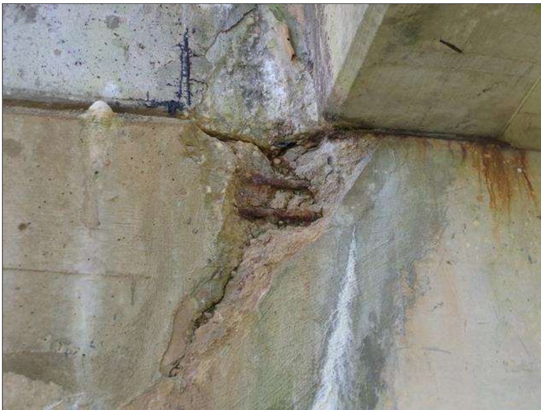
End Bent 1 Abutment/Backwall : 1.5' wide x 2.5' long x 3" deep spall with exposed rebar with no measurable section loss at beam 5.
