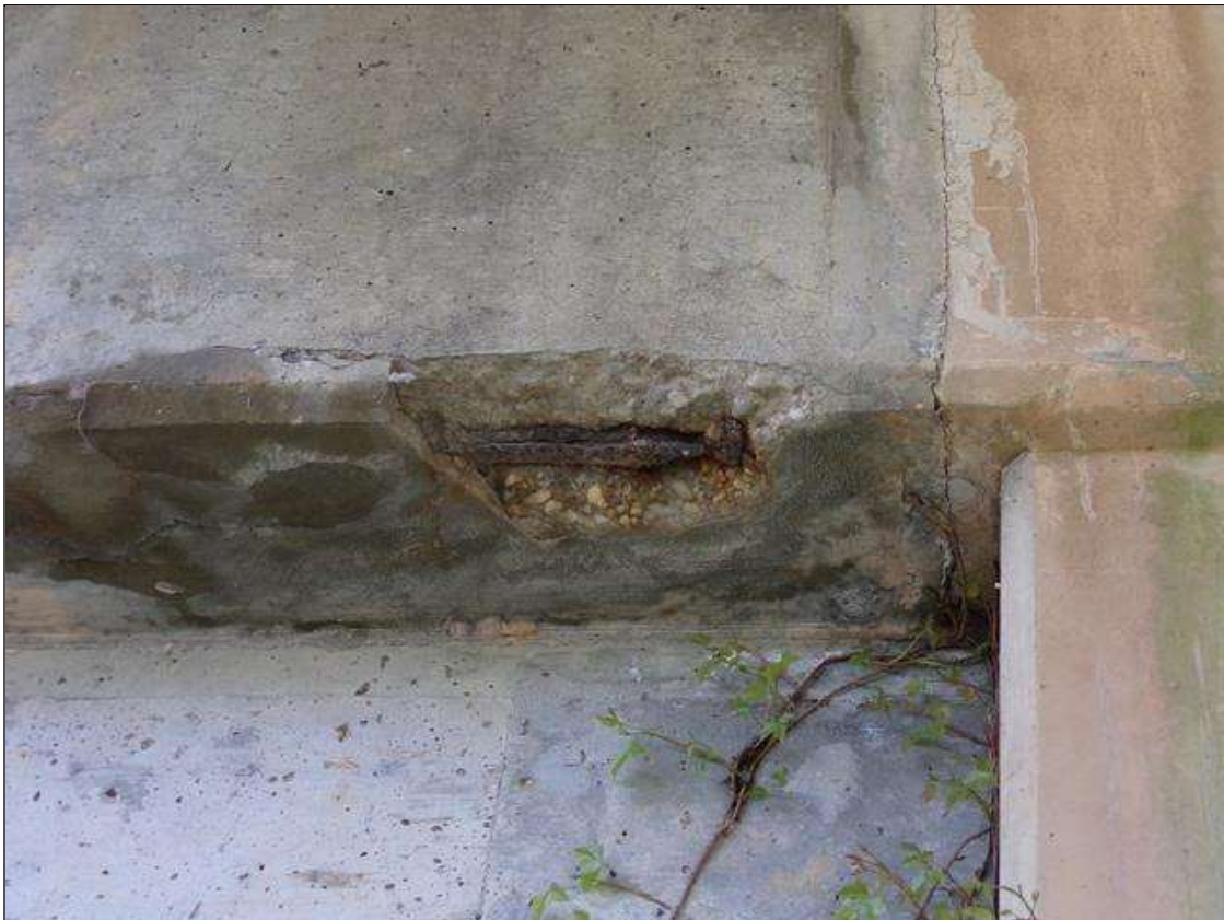
Bent 4 Cap 1: 1' long x 8" wide spall with exposed rebar with no measurable section loss with an area of delamination 1' long x 8" wide next to spall on bottom corner of cap south face between columns 1 and 2.
