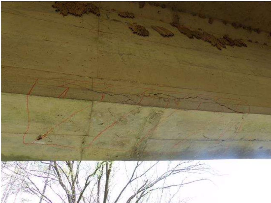
Span 10 Beam 5: Delamination 3' long x 1' wide on bottom of beam x 3" high on west face approximately 10' from pier 9.
