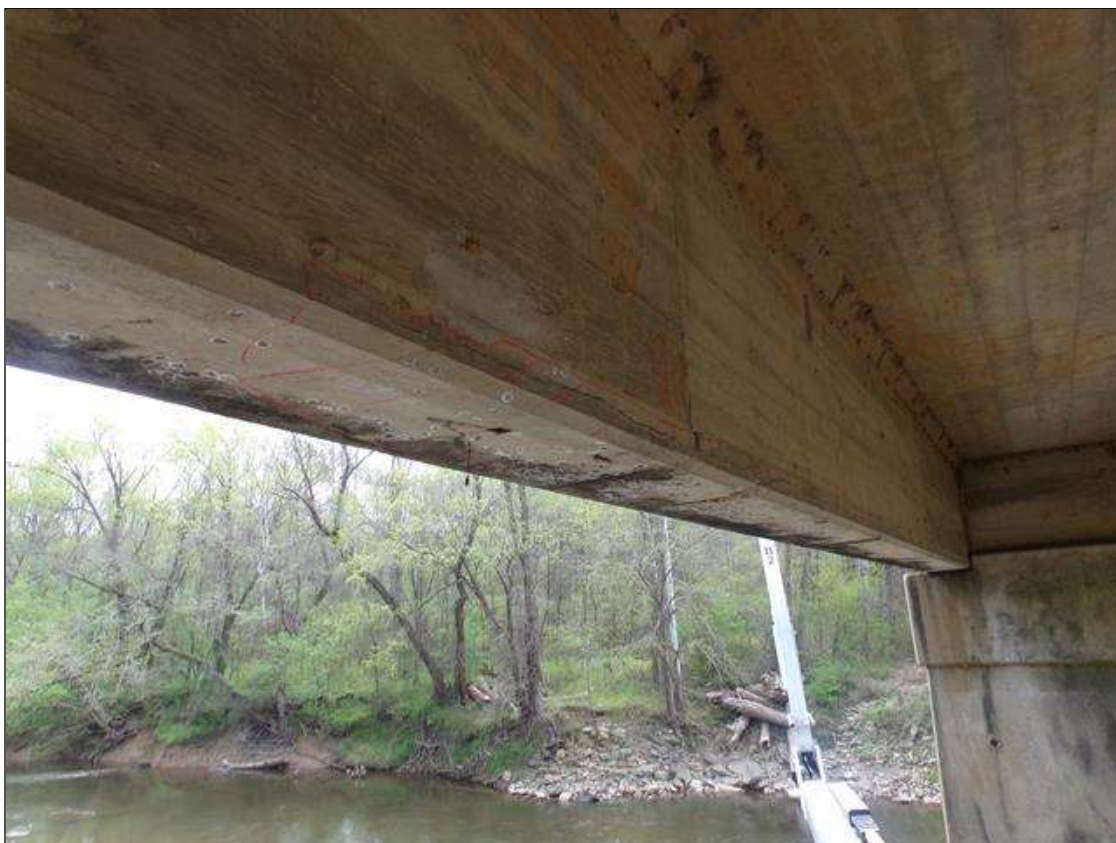
Span 7 Beam 5: Delamination 20' long x up to full width on bottom of beam x 4" high on west face at mid span.
