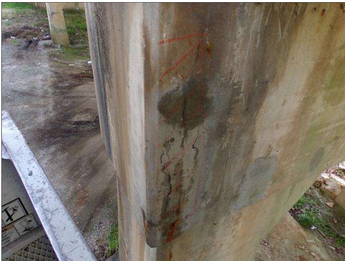
Bent 2 Cap 1: 6" wide x 30" high area of delamination at east end of cap under beam 5
