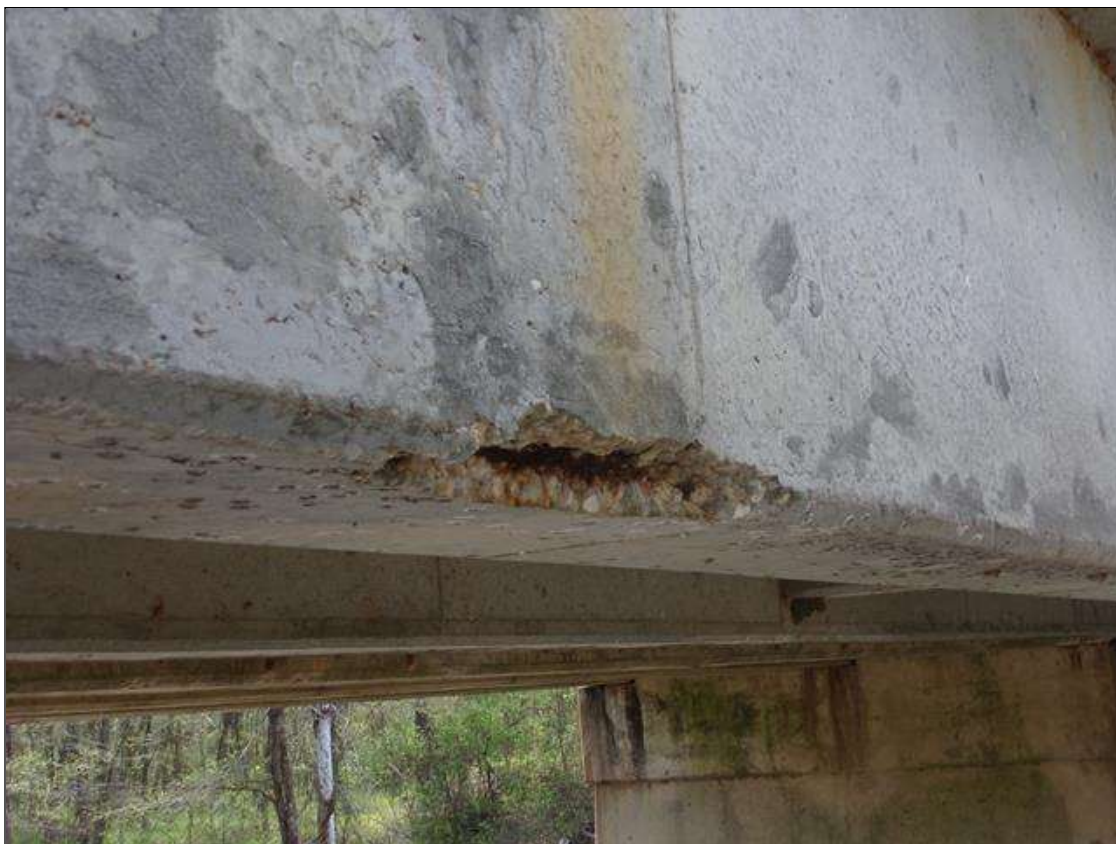
Span 6 Beam 1: 1' long x 4" wide x 1 1/2" deep corner spall with exposed rebar with no measurable section loss on bottom of beam west face 7' from pier 6.
