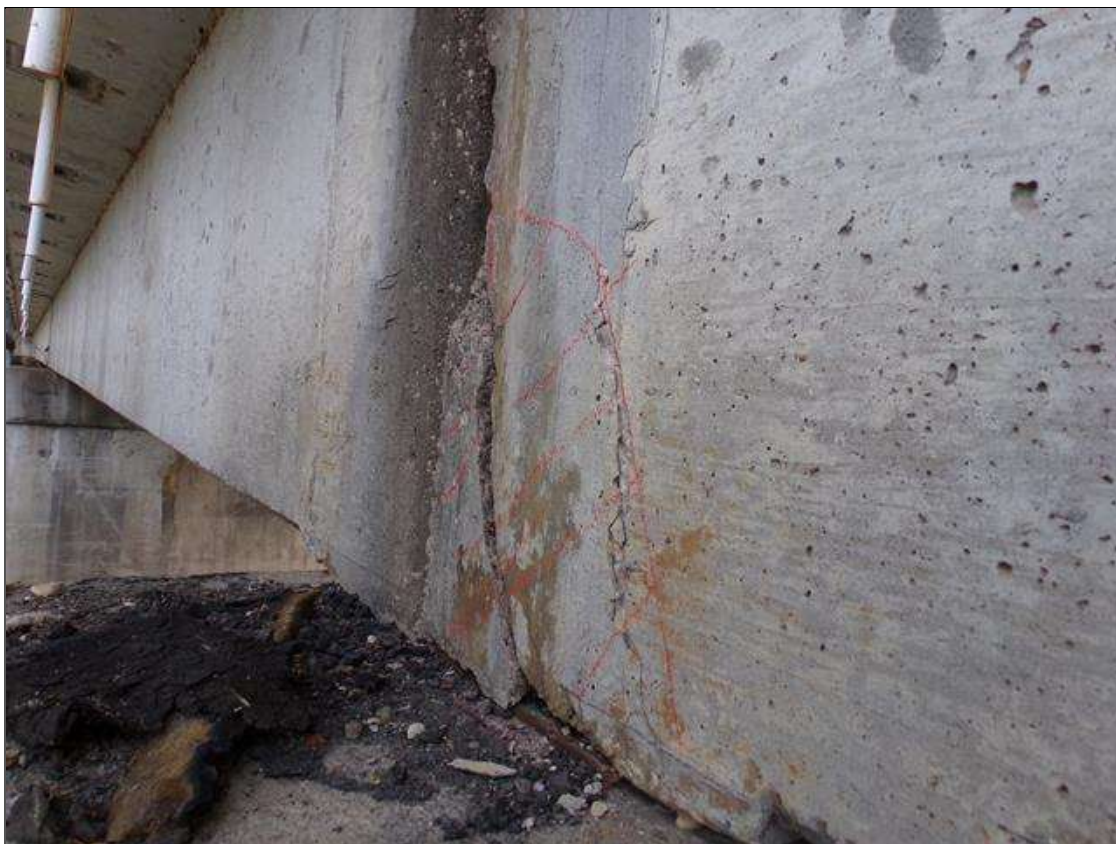
Span 7 Beam 1: Delamination 25" high x 16" wide on west face of beam over pier 7
