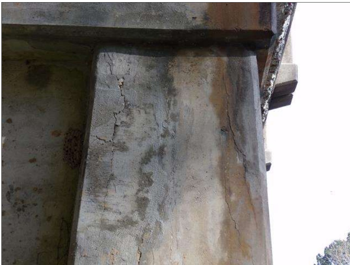
Bent 4 Pile 3: Patched area 4' high x 1' wide on southwest corner and 2' high x 6" wide on southeast corner that are unsound.
