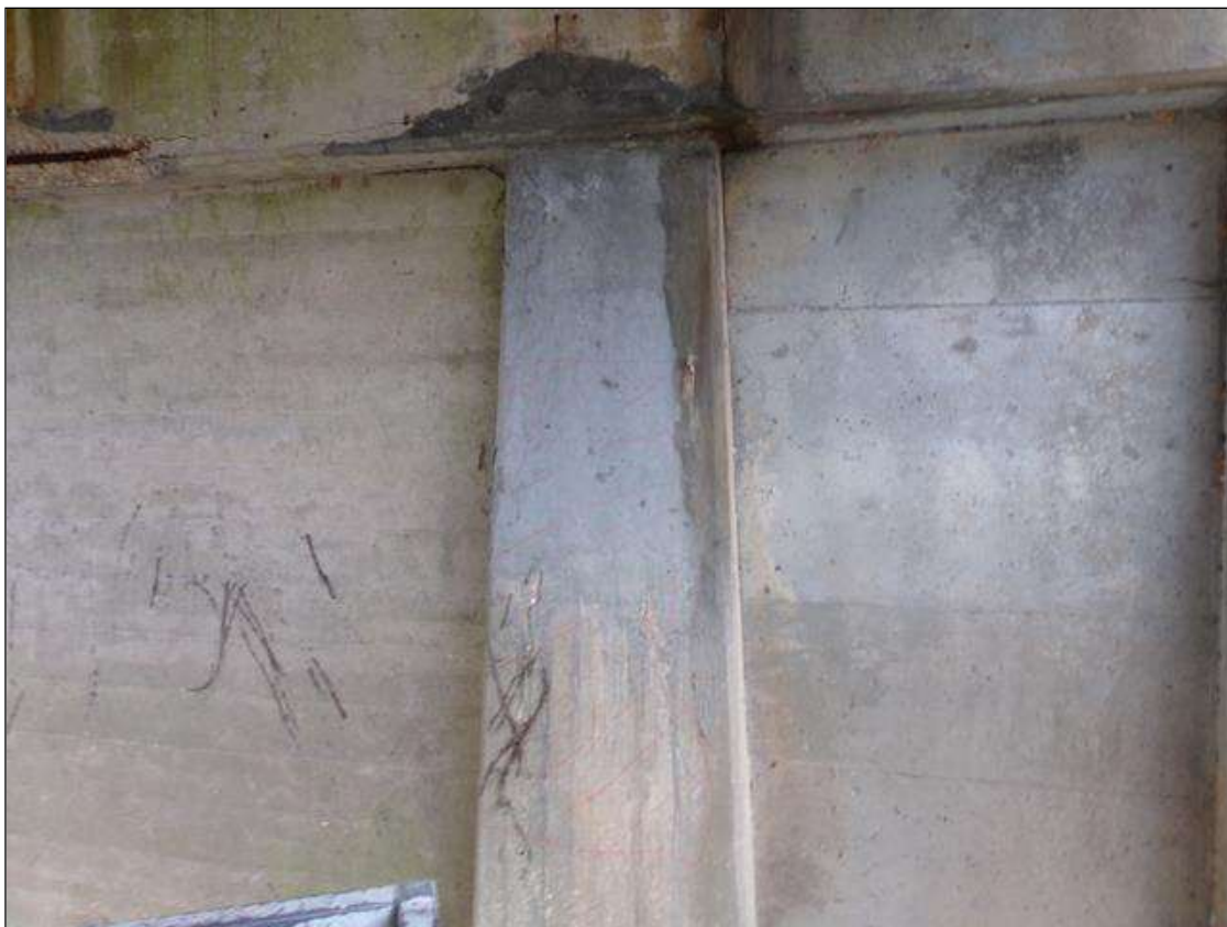
Bent 4 Pile 2: 5' high x 3' wide area of delamination on north face of column starting 3' from bottom of cap.
