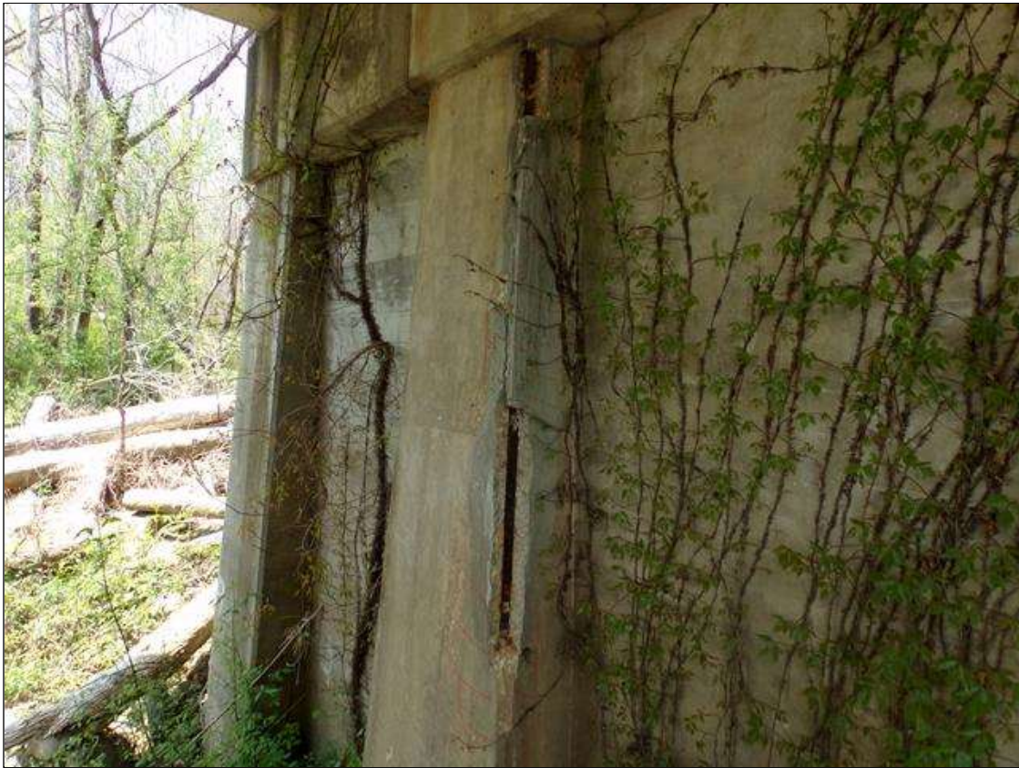
Bent 9 Pile 2: 9' high x up to 1' wide on south face x up to 5" wide on east face delaminated area with 2 spalls up to 3' high x 5" wide x 2" deep with exposed rebar with no measurable section loss starting at bottom of cap.
