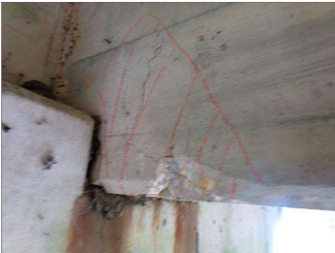
Span 6 Beam 4: Delamination 16" high x 1' long x 9" wide on bottom of beam with a 7" wide x 4" long x 3" deep corner spall at bottom of beam on west face at pier 6.
