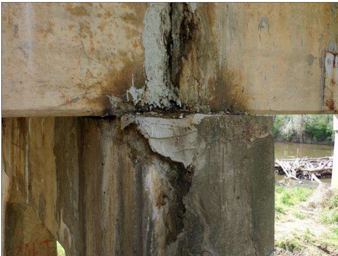
Bent 3 Cap 1: Unsound patched area on top of cap east end with 4" wide x 1/2" deep spalling around patch that extends down east face and south face.
