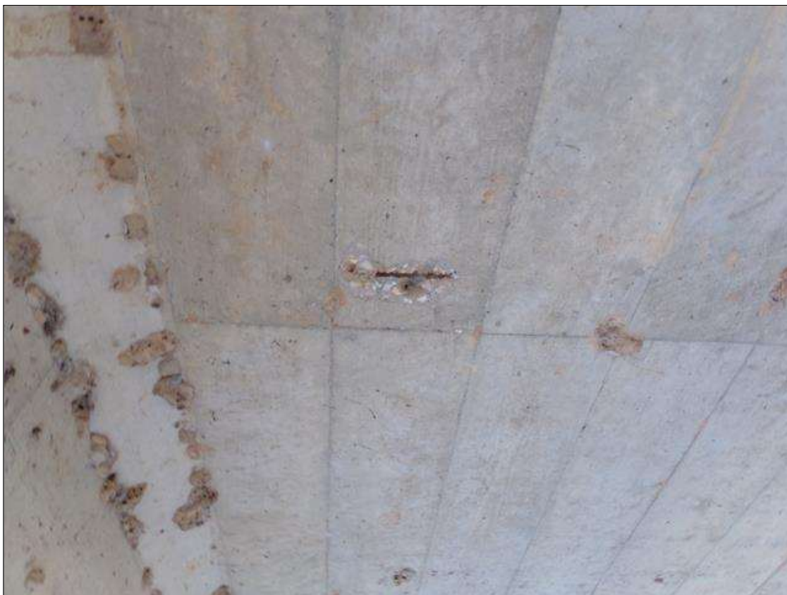
Span 8 Deck: Spall 6" wide x 3" long x 1/4" deep with exposed rebar with no measurable section loss on underside of deck near mid span in bay 3.
