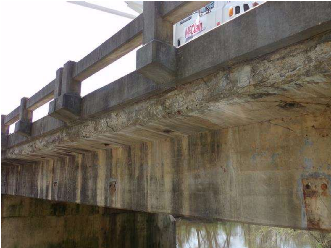
Span 9 Deck: 40' long x full height of front face east overhang area of concrete deterioration with a spalling up to 3" deep throughout starting at pier 9.
