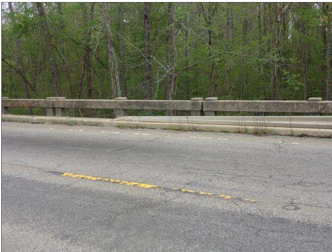
Sand and vegetation accumulation along both curbs blocking drain holes, right curb span 1 shown.
