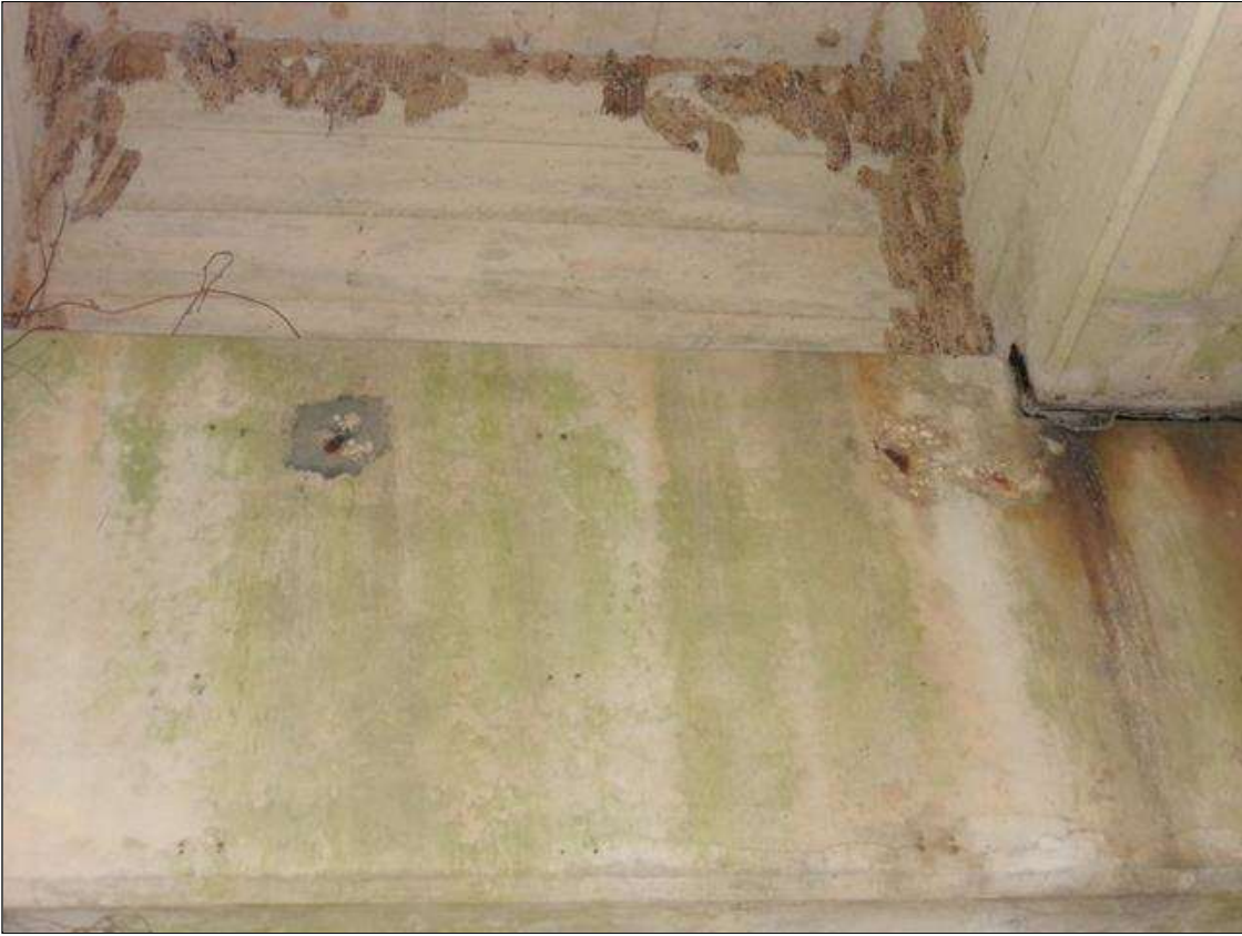
Bent 9 Cap 1: Two spalls up to 6" diameter x 1" deep with exposed rebar with no measurable section loss on north face of cap under bay 3.
