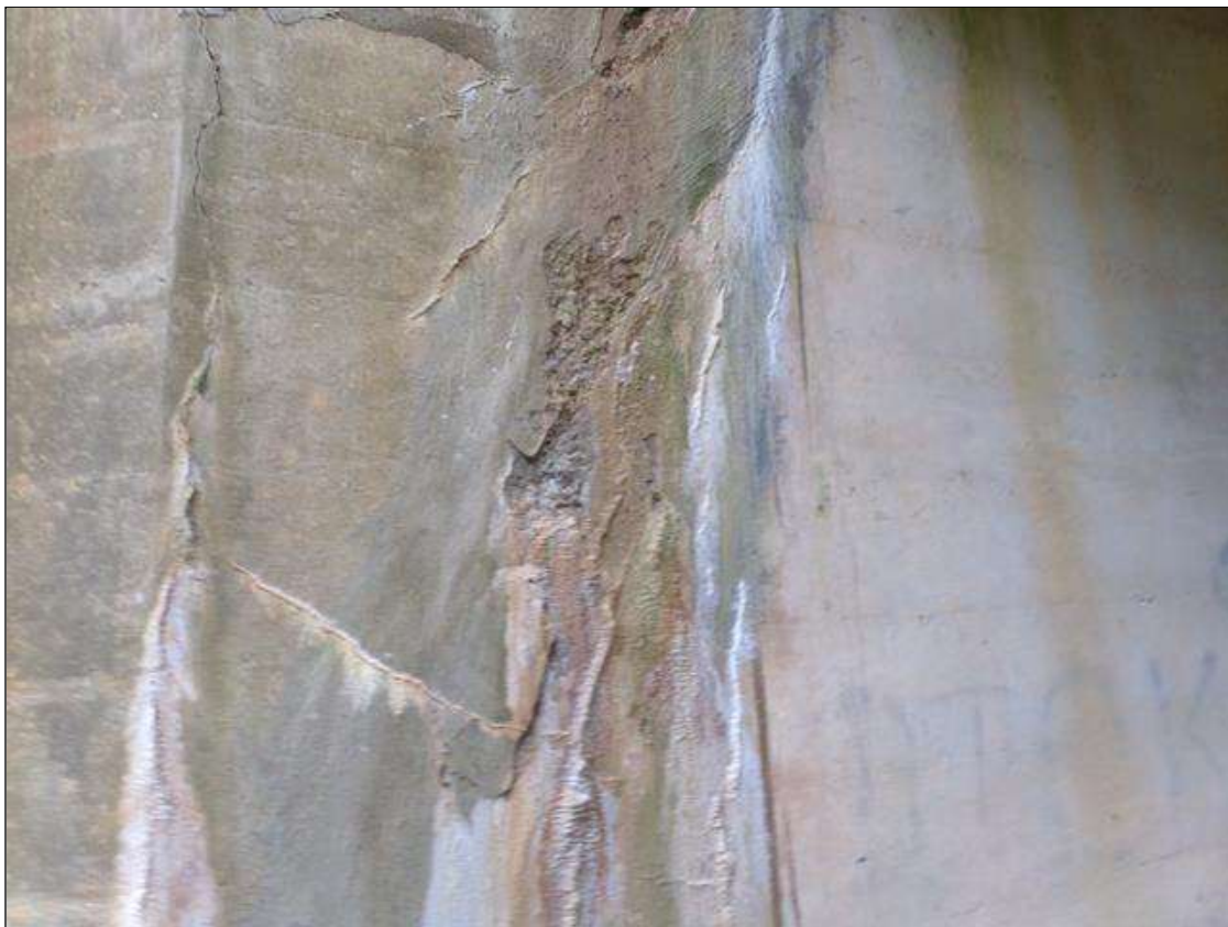
End Bent 1 Abutment/Backwall : Patched area that is unsound 16" wide x 5' high on front face under beam 5.
