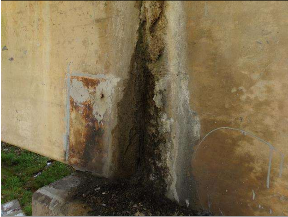
Span 2 Beam 5: 18" high x 4" wide x 1" deep spall on east face of beam over pier 1
