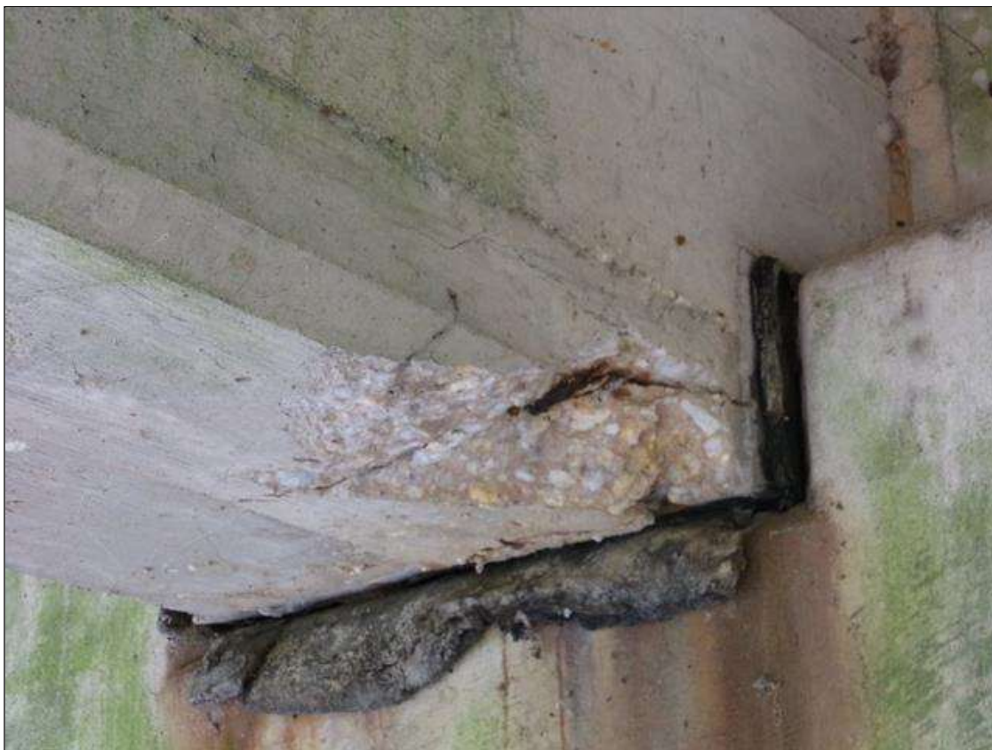
Span 7 Beam 4: 10" long x 6" wide x 1" deep spall with exposed rebar with no measurable section loss on bottom of beam at pier 6
