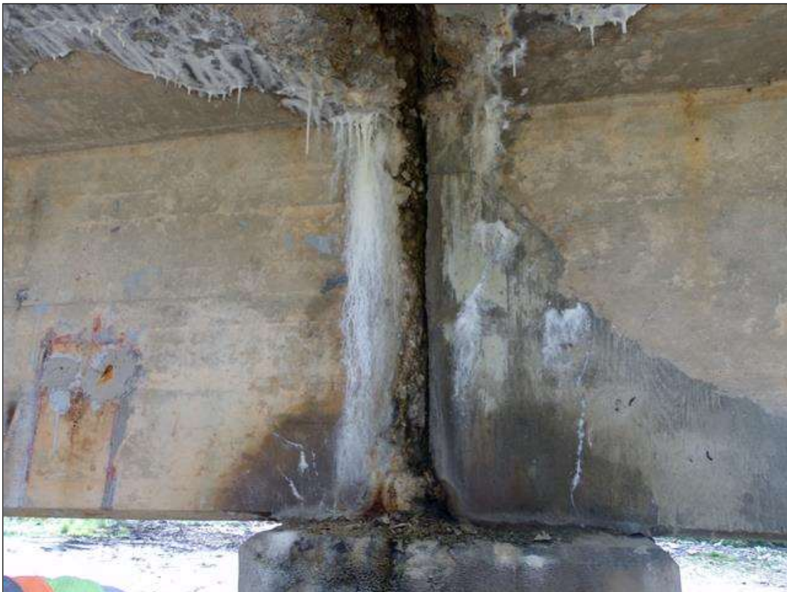
Span 2 Beam 5: Full height x 3" wide x up to 1" deep spall at end of beam over pier 2 east face.
