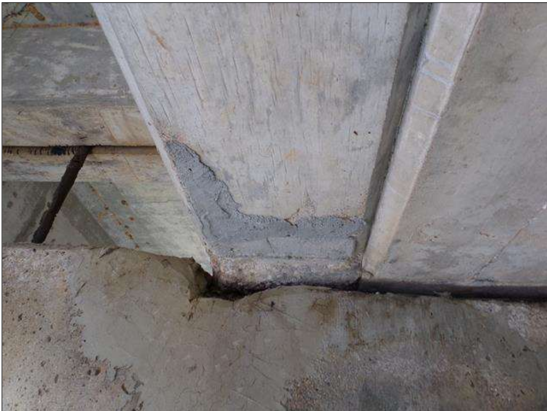
Span 2 Beam 2: 10" long x full width of bottom of beam sound patched area at pier 2.
