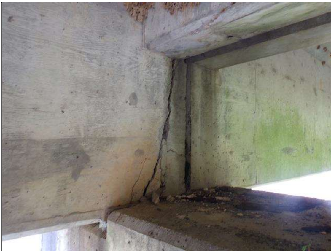
Span 9 Beam 1: Spall at beam end 1' wide x 26" high x full width over pier 9
