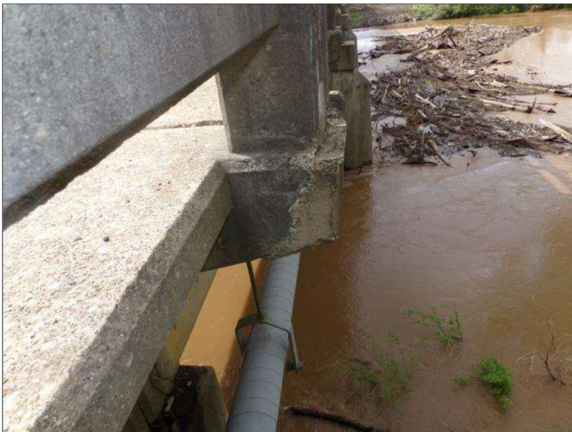
Span 10 Left Bridge Rail: Sound patched area on bottom west face of rail post 1.
