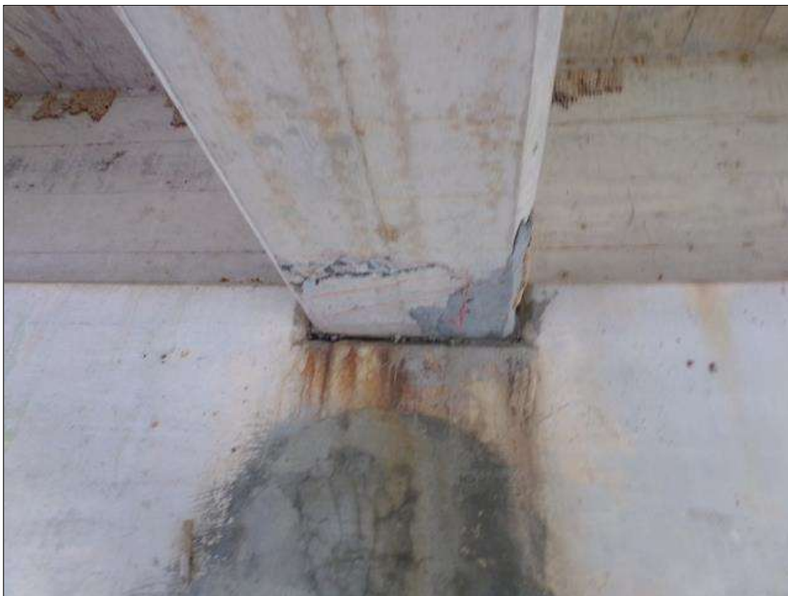
Span 3 Beam 4: 1' square area of delamination with a 10" long x 3" wide x 1/2" deep spall on bottom of beam at pier 2.
