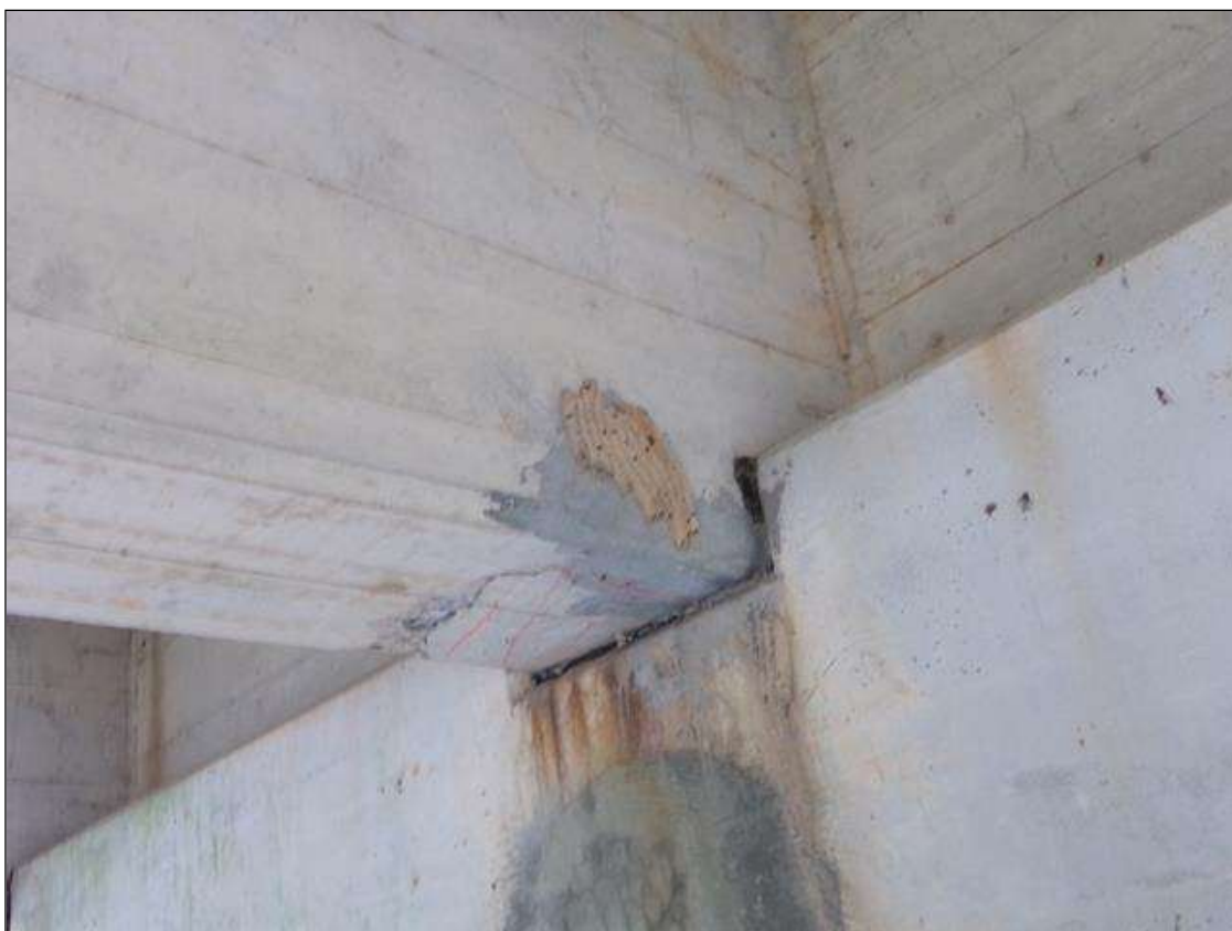
Span 3 Beam 4: Sound patched area 1' long x 3" high on west face x 6" wide on bottom of beam at pier 2.
