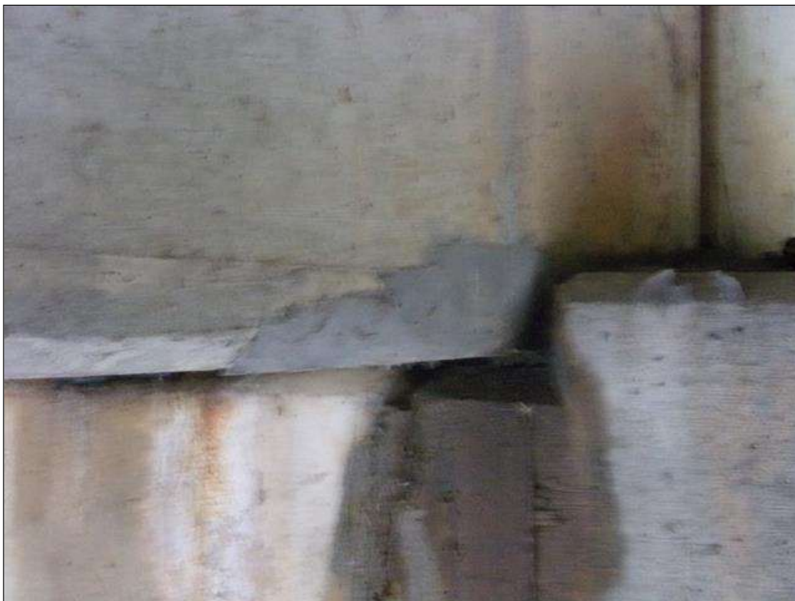
Span 5 Beam 2: 18" long x 4" high on west face x 4" wide on bottom of beam sound patched area starting at pier 4.
