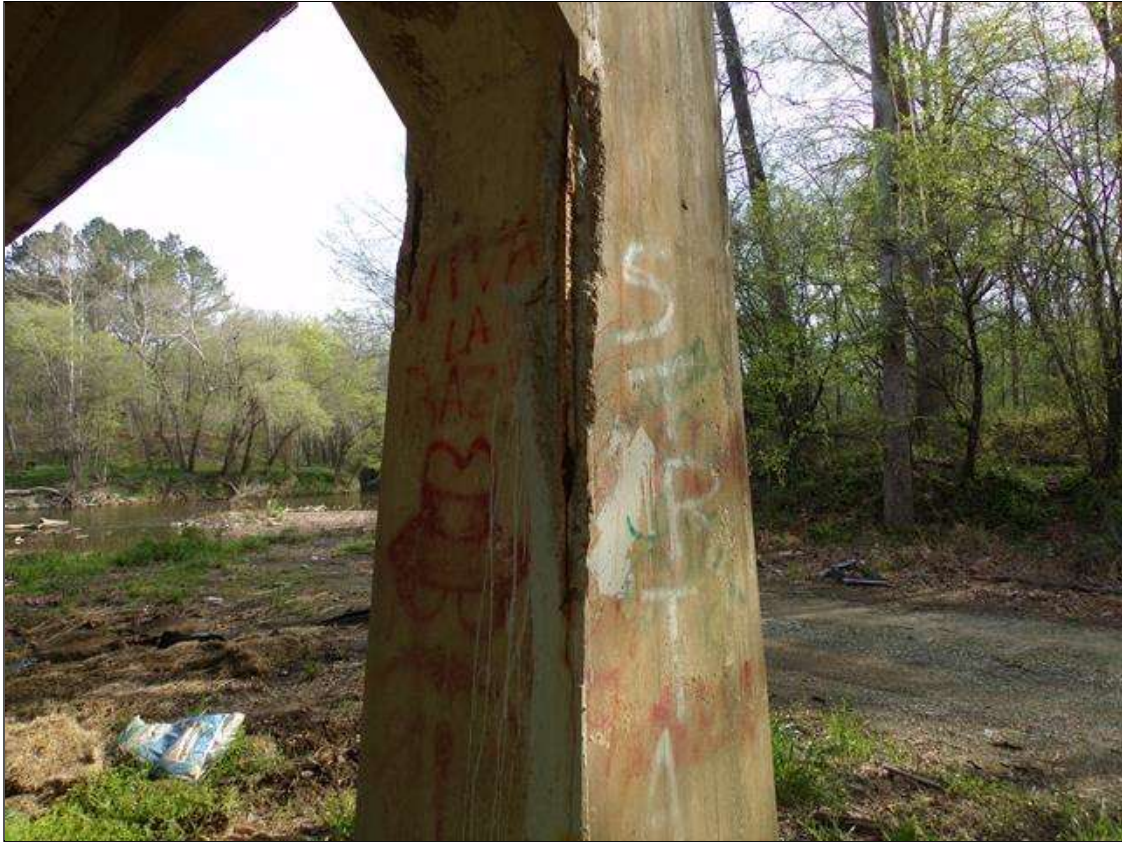
Bent 3 Pile 3: 5' high x 8" wide corner spall with exposed rebar with no measurable section loss on southwest corner with areas of delamination on both sides of spall with a crack up to 1/8" wide that extends down to ground starting 2' from bottom of cap.
