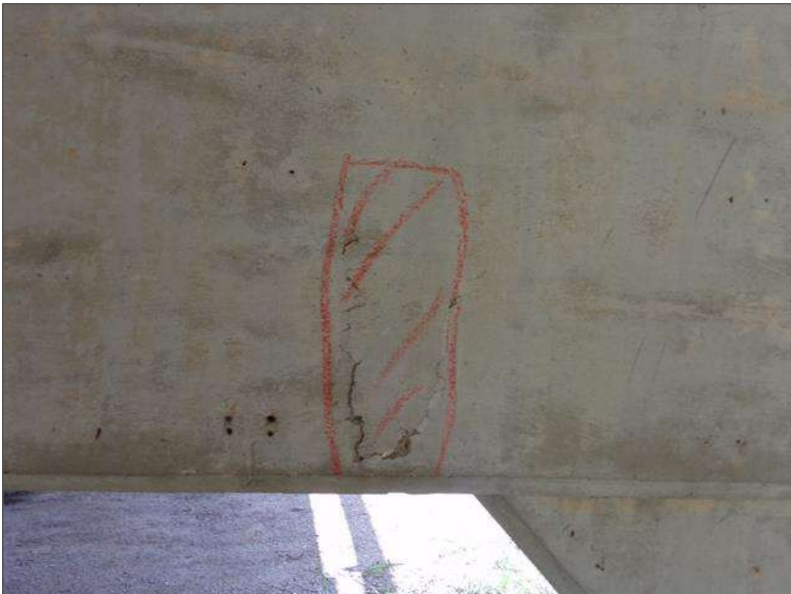
Bent 2 Cap 1: 6" wide x 11" high area of delamination on north face of cap under bay 2.
