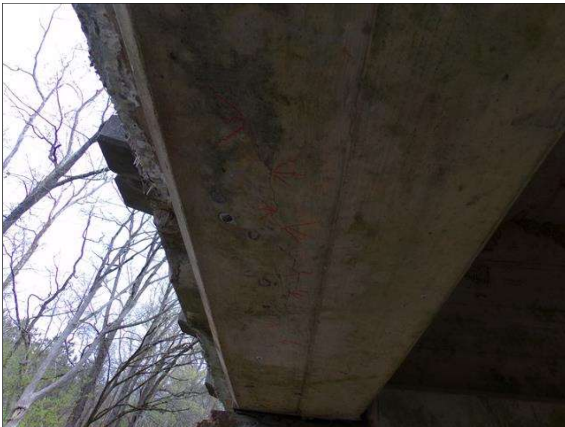
Span 5 Beam 5: 2' long x 1/32" wide longitudinal crack on bottom of beam starting 2' from pier 4.
