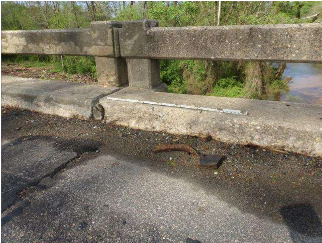
Span 5 Left Bridge Rail: 4' long x up to full height x up to 1" deep spalled area on front face of curb starting at pier 4
