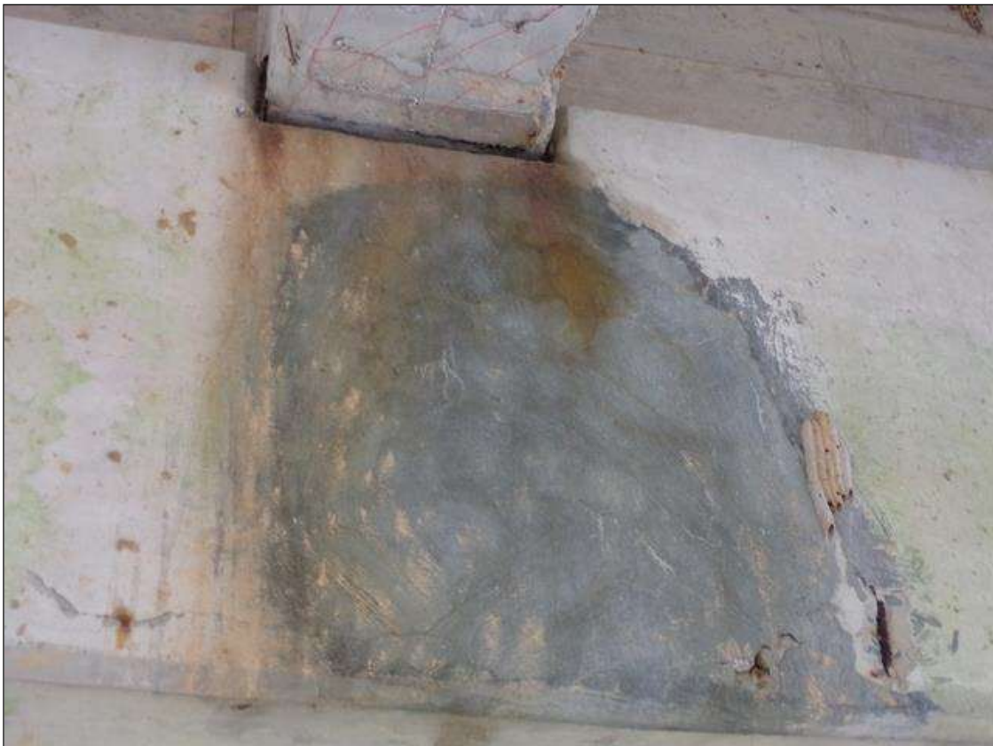
Bent 1 Cap 1: 3' high x 2' wide unsound patched area with on north face of cap with 2 spalls up to 4" diameter 1/2" deep with exposed rebar with no measurable section loss under beam 4.
