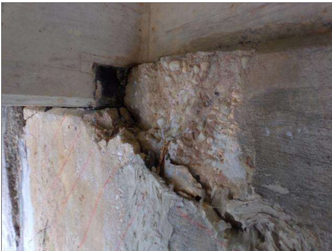
Bent 3 Cap 1: 1' high x up to 19" wide x up to 5" deep spall on south face of cap under bay 2
