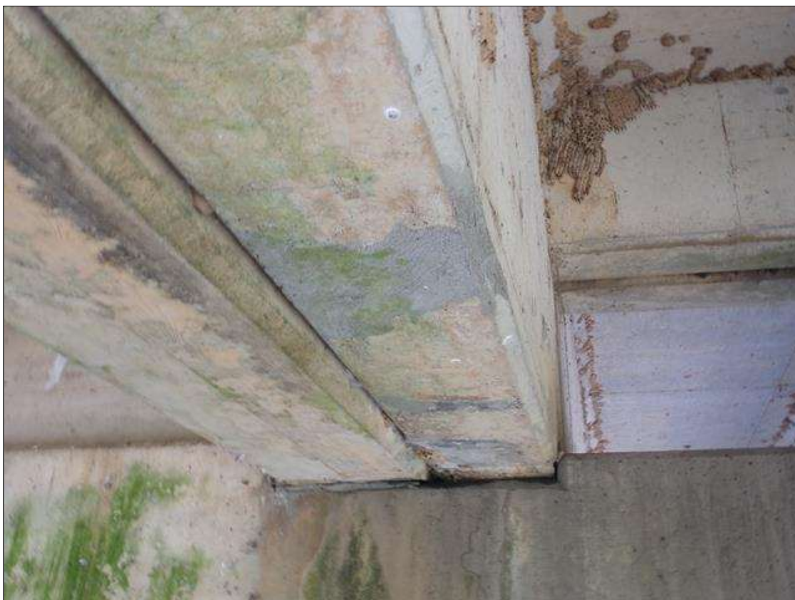
Span 9 Beam 2: Three sound patched area on bottom of beam up to 1' wide x 10" long starting at pier 8 out 4'.
