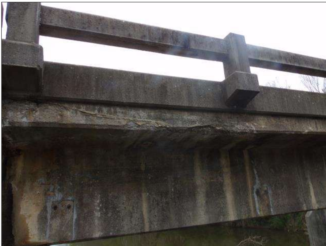
Span 6 Deck: 15' long x full height of front face east overhang area of concrete deterioration with a spall 2' long x 7" wide x up to 2" deep starting at pier 5.
