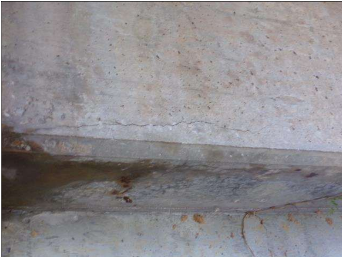
Bent 1 Cap 1: 2' long horizontal/transverse crack up to 1/16" wide on north face and bottom of cap starting at construction joint.
