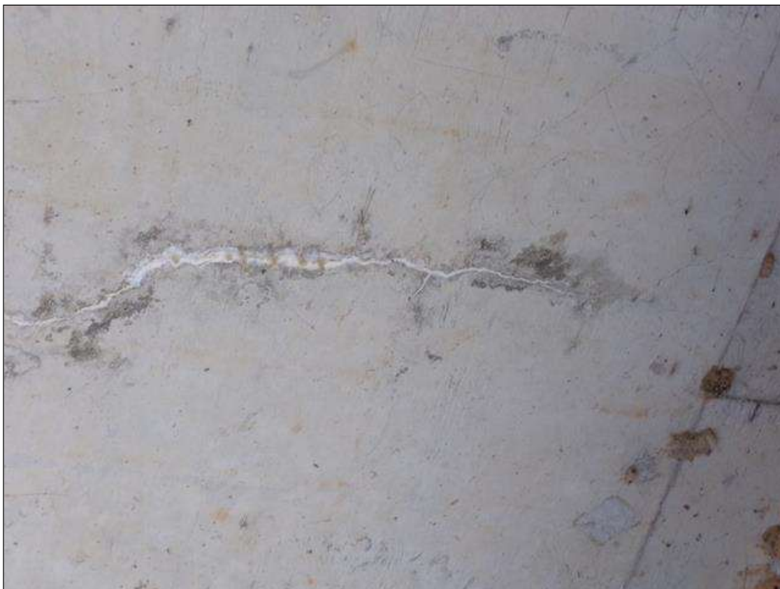
Span 9 Deck: Full width hairline transverse crack with efflorescence and stalactites on underside of deck 5' from pier 9 in bay 1.
