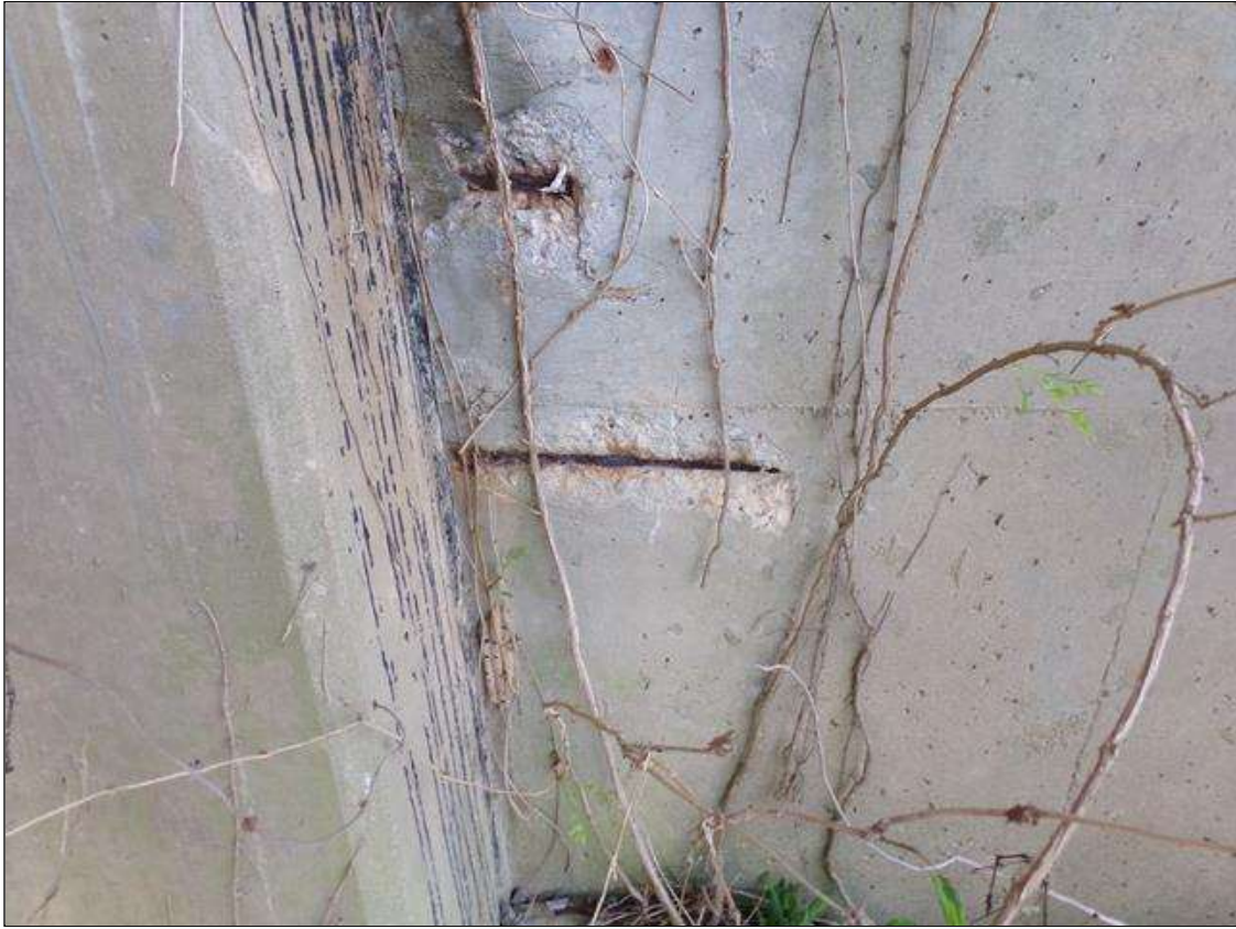
Two spalls up to 16" long x 4" wide x 1/2" deep with exposed rebar with no measurable section loss on north face of web wall next to column 2
