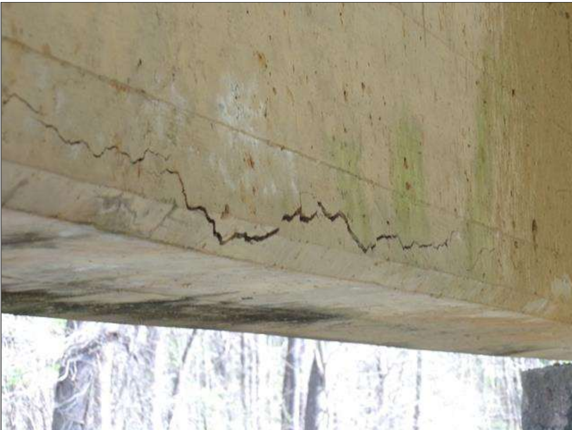
Span 4 Beam 5: 15' long x up to 1/4" deep horizontal crack in west face 1" up from bottom of beam at mid span.
