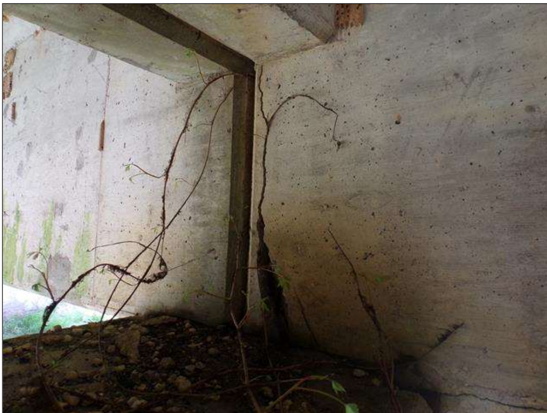
Span 9 Beam 2: Spall at beam end west face 3" wide x 10" high x 1 1/2" deep with a 16" long vertical crack 1/4" wide over pier 9
