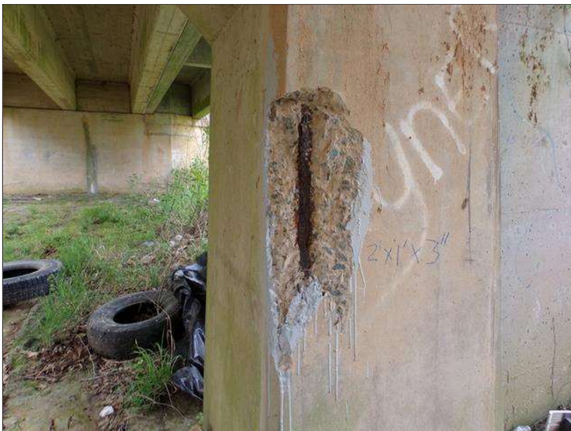
Bent 1 Pile 2: PM--2' high x 1' wide x 3" deep spall with exposed rebar with section loss on north face starting 3' from ground line.
