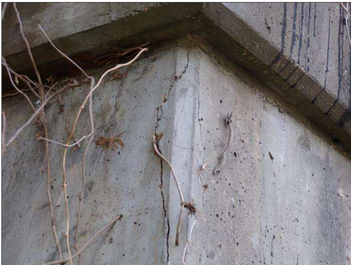
Bent 2 Pile 1: 2' long x 4" wide area of delamination on northwest corner starting at bottom of cap.
