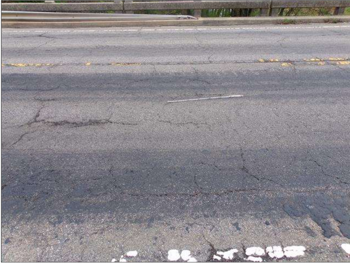
Span 10 Wearing Surface: Transverse/longitudinal/map cracking in AWS up to 1/2" wide throughout span both travel lanes.
