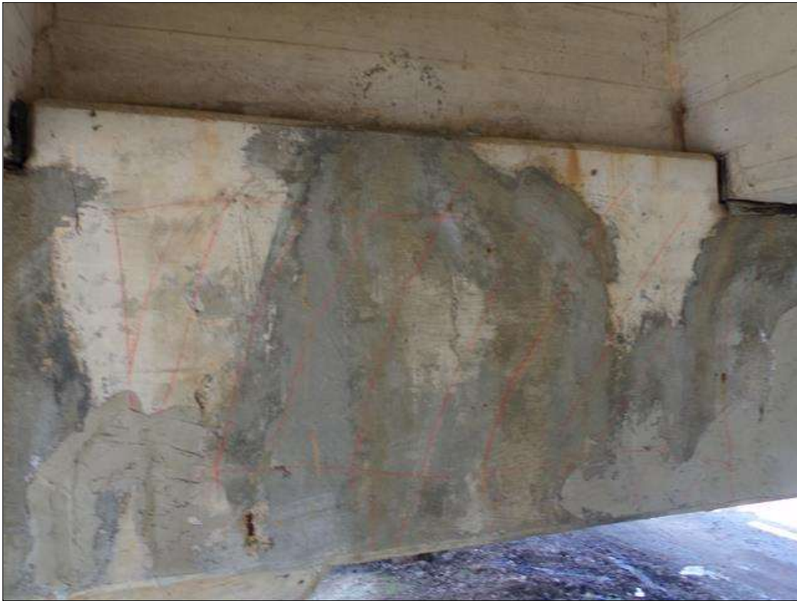
Bent 2 Cap 1: Delamination 3' high x 6' long on south face of cap under bay 2.
