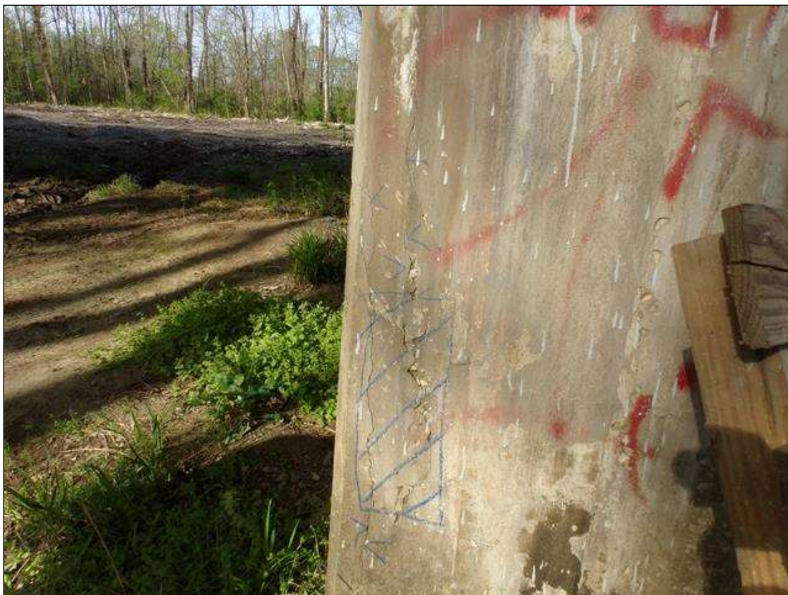
Bent 3 Pile 3: 1.5' high x 6" wide area of delamination with 1/32" cracks that extend 2' up and down from delamination.
