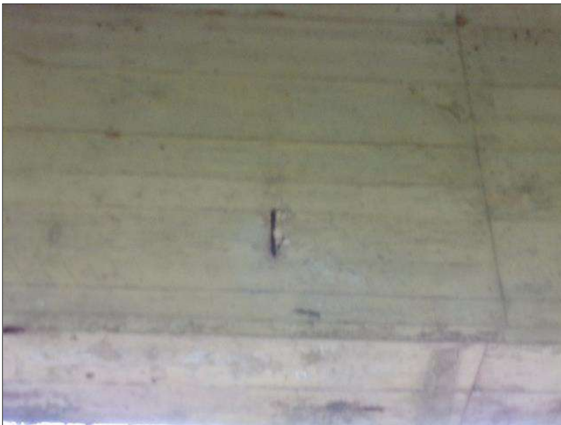
Span 1 Beam 5: 6" high x 2" wide x 1/4" deep spall with exposed rebar with no measurable section loss on west face of beam near mid span.
