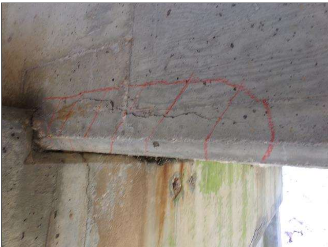
Span 4 Beam 2: Area of delamination 20" long x 5" high on west face x 5" wide on bottom of beam at pier 4.
