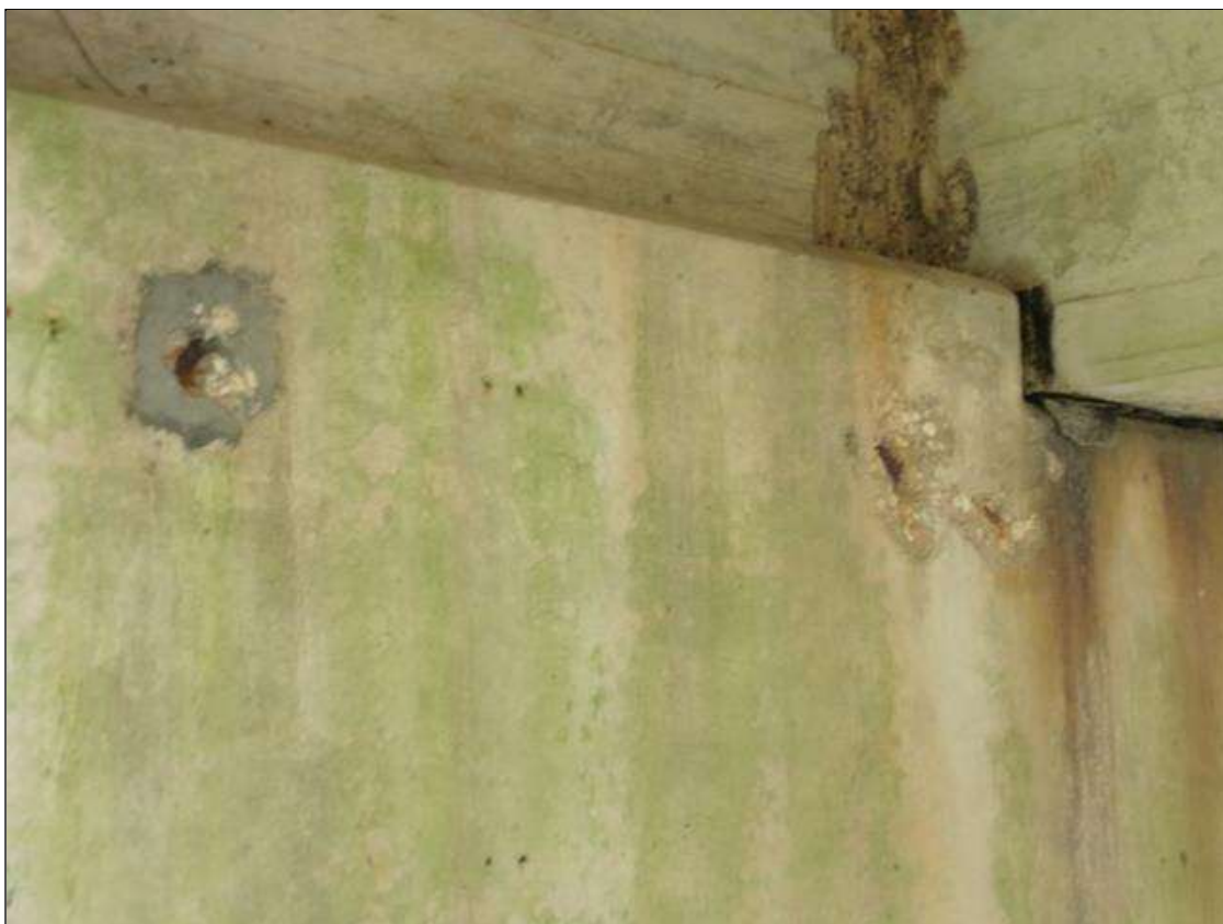
Bent 9 Cap 1: Three spalls up to 8" diameter x 3/4" deep with exposed rebar with no measurable section loss on north face of cap under bay 3
