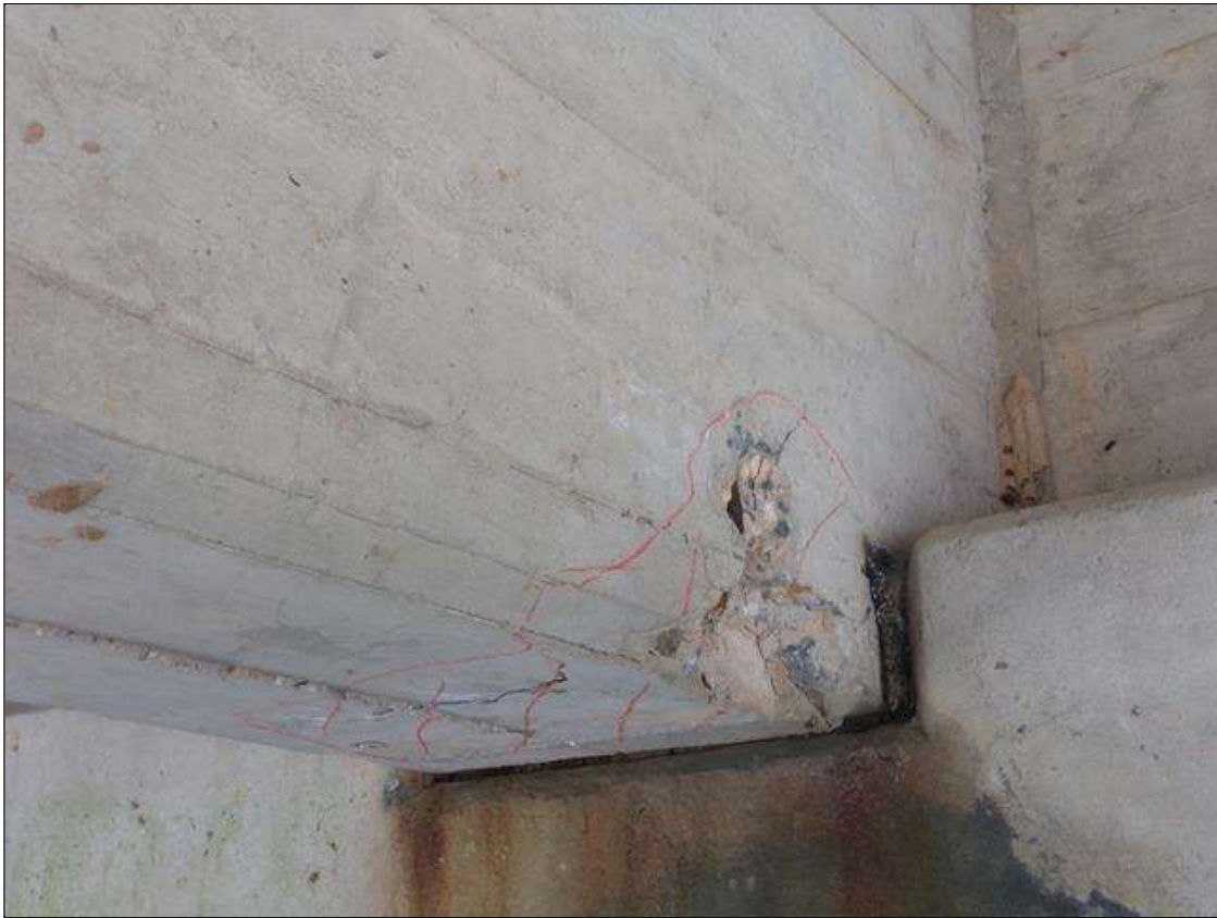
Span 2 Beam 4: Area of delamination 1' square on bottom of beam x 1' high on west face with a spall 6" high x 6" with x 1" deep with exposed rebar with no measurable section loss at pier 1.
