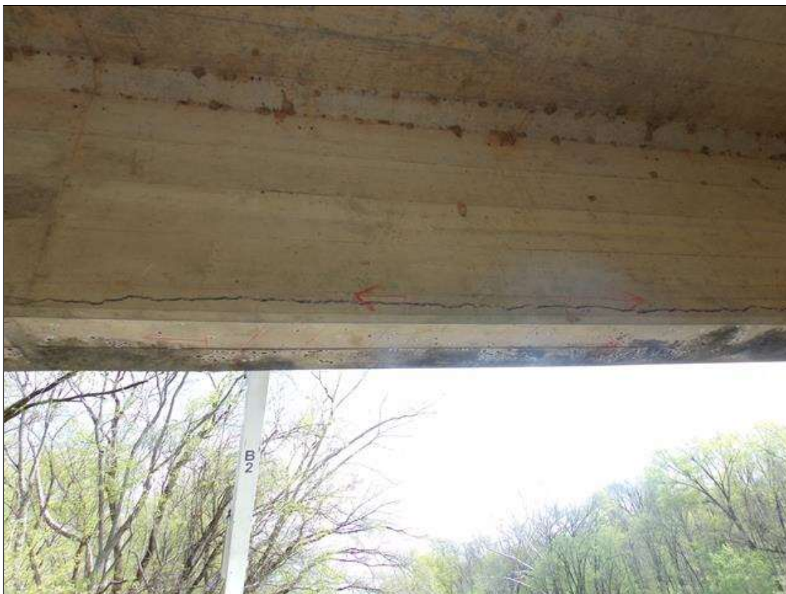
Span 9 Beam 5: Delamination 30' long x up to full width of bottom of beam x up to 1' on west face starting approximately 10' from pier 9.
