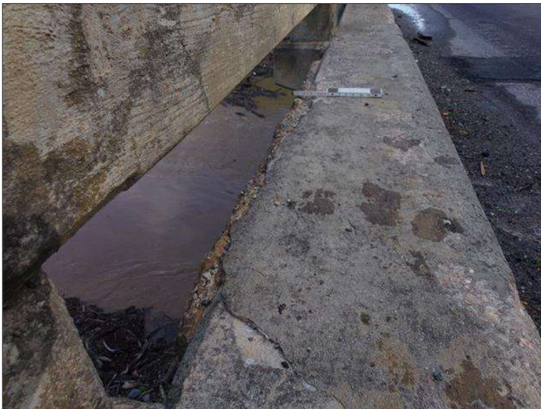
Span 4 Left Bridge Rail: unsound patched area on west face of curb between rail posts 8 and 9.
