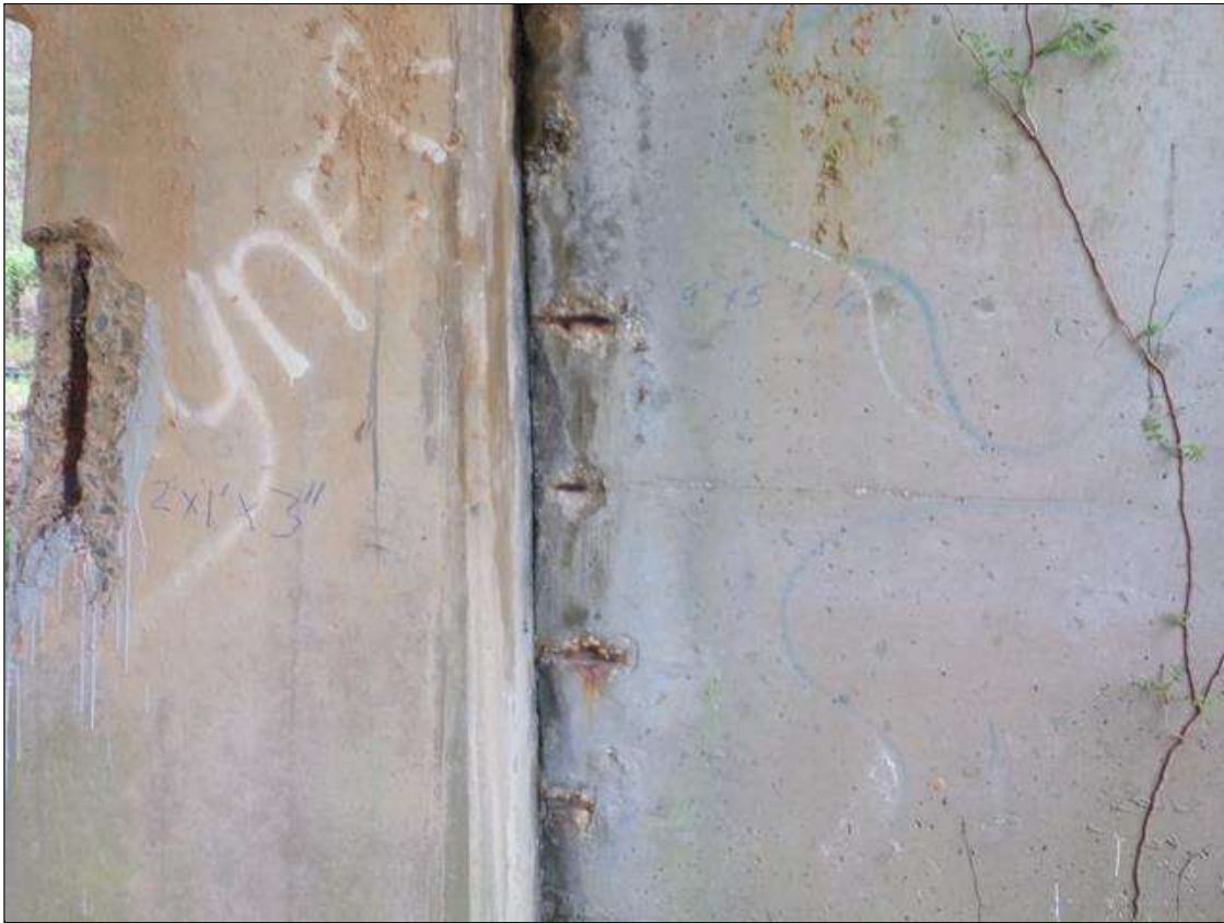
Several spalls up to 8" wide x 6" long x 1/2" deep with exposed rebar with no measurable section loss on web wall next to column 2 north face.
