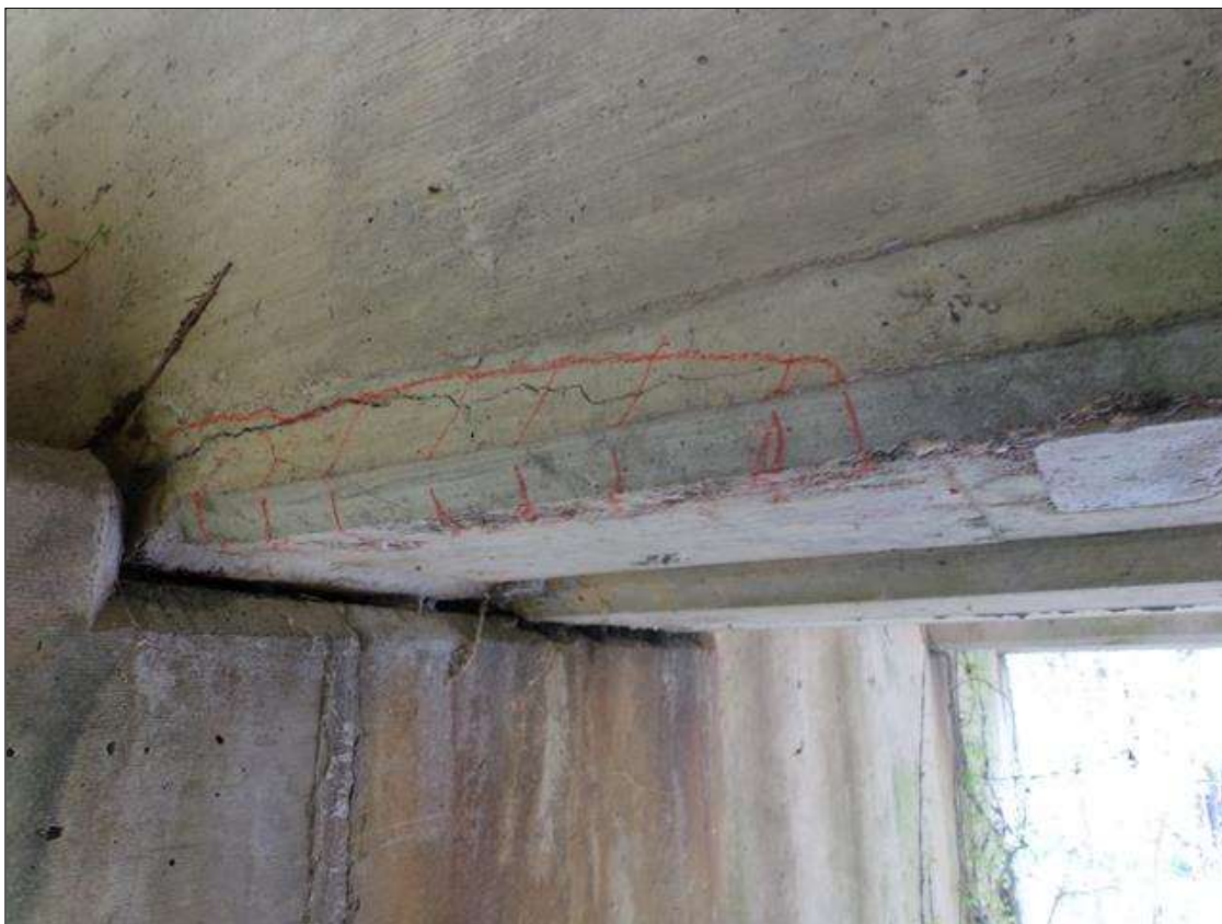
Span 9 Beam 2: Delamination 16" long x 3" high on west face x 4" wide on bottom of beam starting at pier 9.
