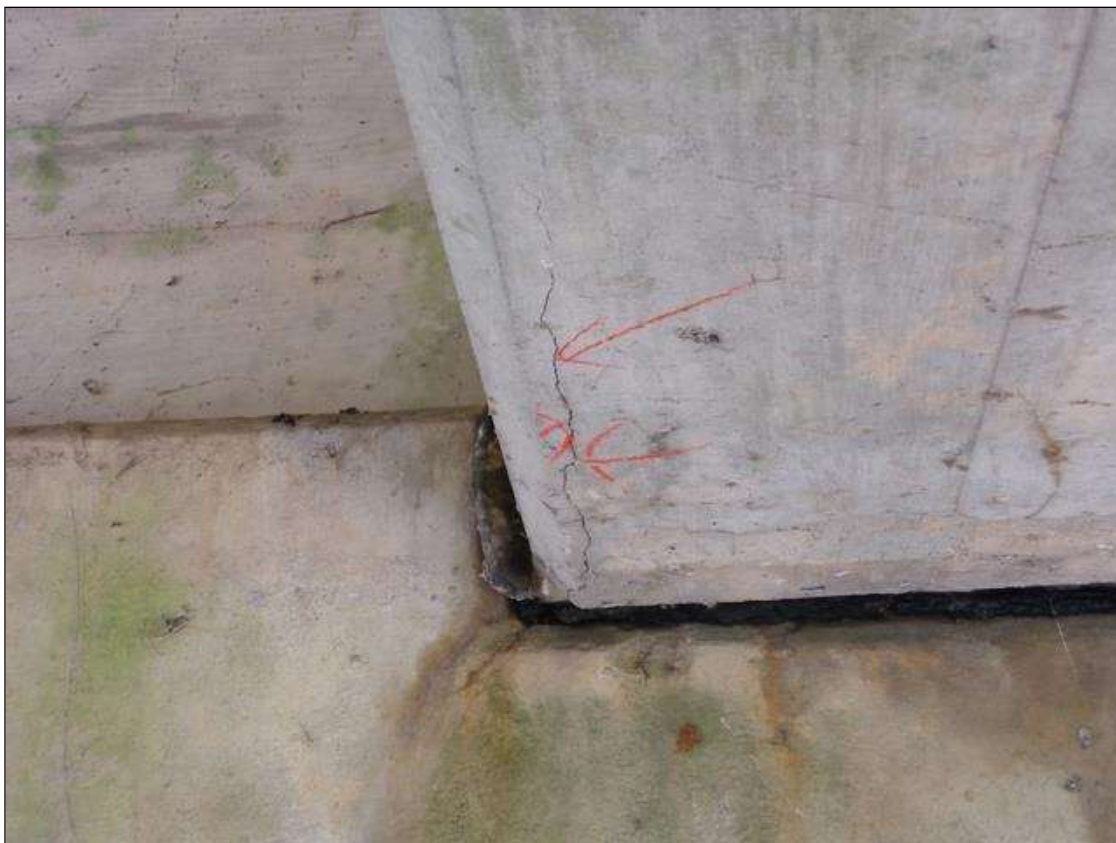
Span 7 Beam 3: 1' long longitudinal crack 1/8" wide on bottom of beam starting at pier 6.
