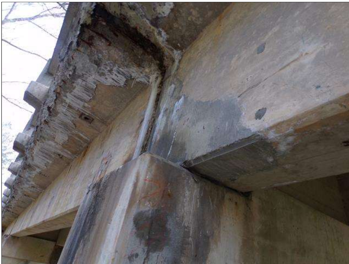
Span 3 Beam 5: Sound patched area full height at end of beam x 3' long at bottom of beam that extends 8" on bottom of beam at pier 2.
