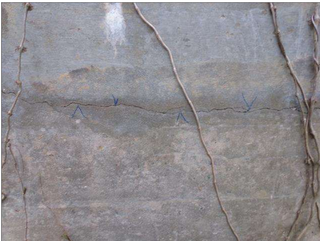
End Bent 1 Abutment/Backwall : 25' long horizontal crack up to 1/8" wide at west end of abutment that extends 3' on front face starting under bay 1.
