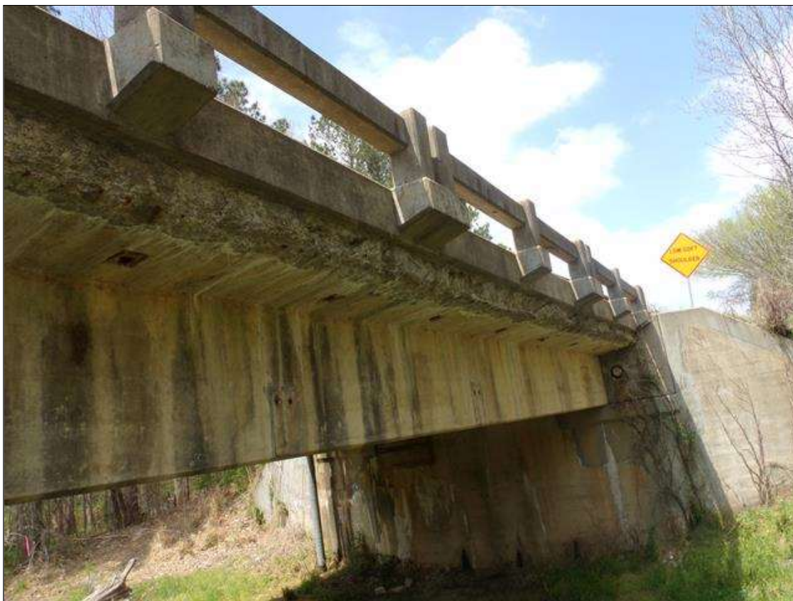
Span 10 Deck: Full length x full height of front face east overhang area of concrete deterioration with a spalling up to 3" deep throughout starting at pier 9.
