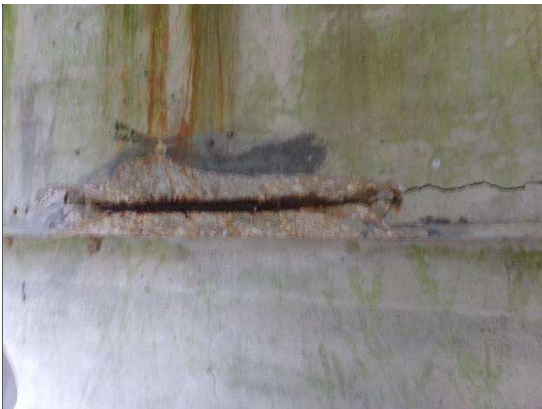
Bent 4 Cap 1: PM--3' long x up to 1' high x up to 5" deep spall on bottom corner of cap with exposed rebar with section loss on north face with a 5' long x 5" high area of delamination.
