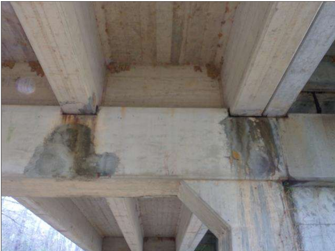
Bent 2 Cap 1: 2 sound patched area on north face of cap under beams 3 and 4.
