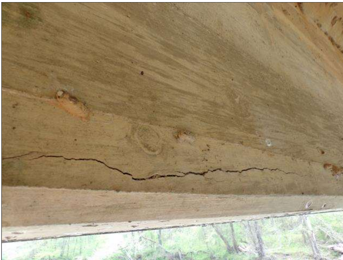
Span 7 Beam 5: 2' long horizontal crack 1/8" wide on west face of beam 16' from pier 7.
