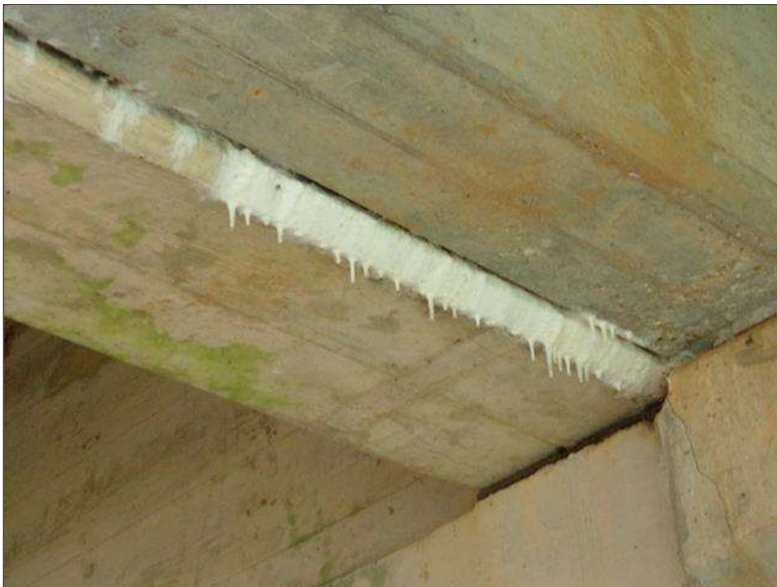
Span 1 Beam 3: 4' of efflorescence on bottom of beam between beams 2 and 3 starting at abutment 1.
