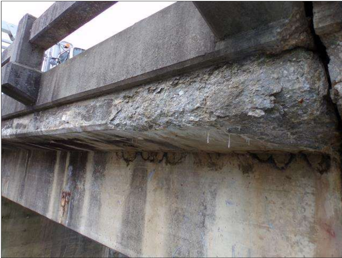
Span 6 Deck: 15' long x full height of front face east overhang area of concrete deterioration with a spall 2' long x 7" wide x up to 2" deep starting at pier 6.
