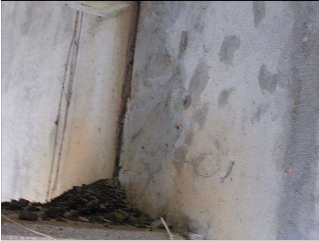
Span 3 Beam 1: 1' wide x 20" high sound patched area on east face of beam over pier 2.
