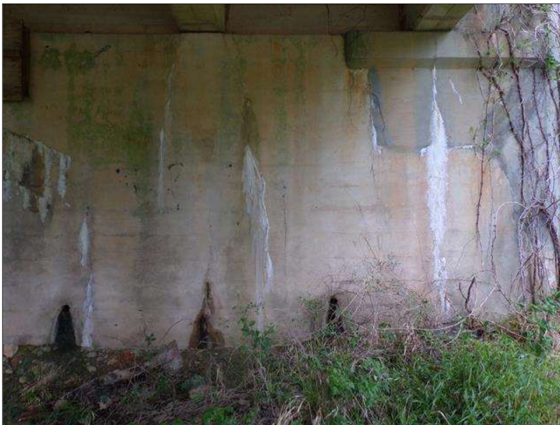
End Bent 2 Abutment/Backwall : Several full/partial height vertical cracks up to 1/16" wide with efflorescence under bay 2 out to beam 5.
