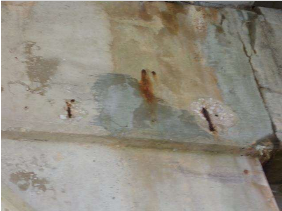
Bent 3 Cap 1: Two spalls up to 6" diameter x 1/2" deep with exposed rebar with no measurable section loss on north face of cap under beam 3.
