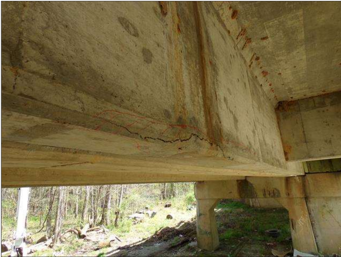
Span 2 Beam 2: Delamination 6' long x 8" wide on bottom of beam x 5" high on west face 9' from pier 2.
