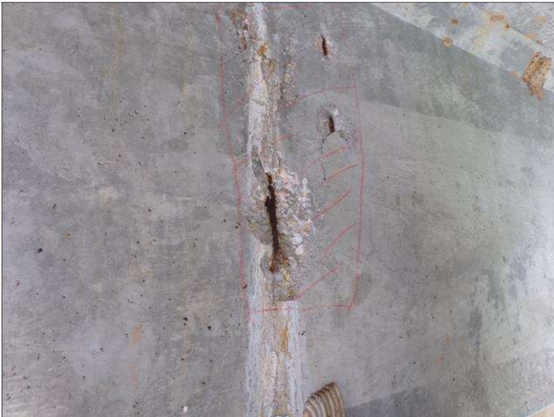
Span 2 Beam 2: 3' high x 16" wide area of delamination on west face of cap 7' from pier 1 with spalls up to 8" long x 6" wide x 1" deep .
