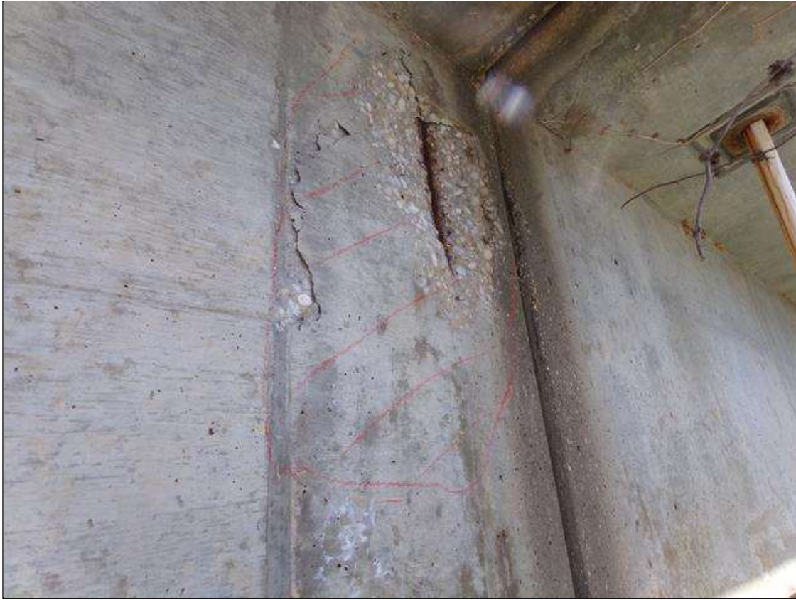
Span 2 Beam 1: 3' high x 2' wide area of delamination on west face of beam with a 16" square x 1" deep spall with exposed rebar with no measurable section loss over pier 1.
