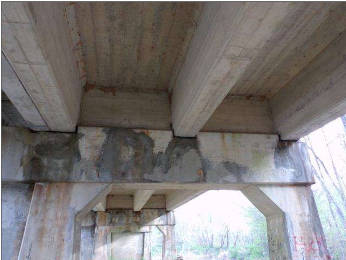
Bent 2 Cap 1: Several sound patched areas on south face of cap between beams 2 thru 5.
