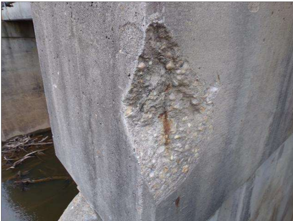
Bent 5 Cap 1: 18" high x 11" wide x 3" deep spall on south face of cap at west end.
