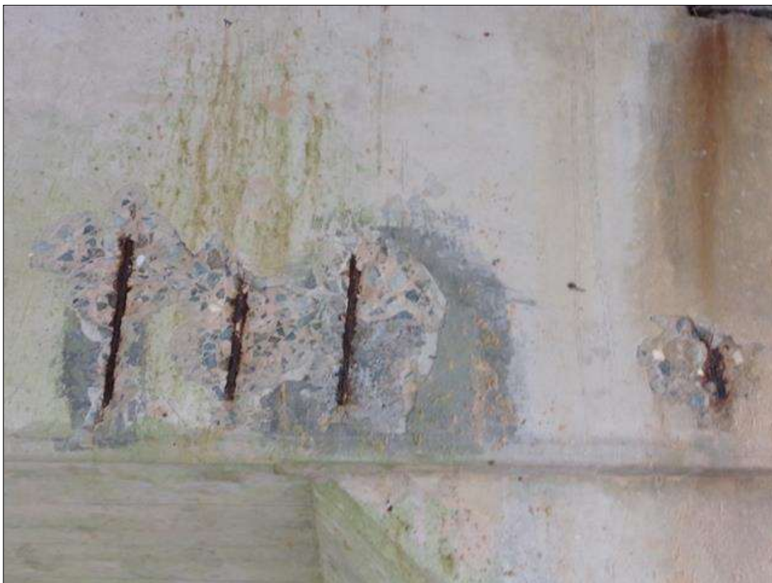
Bent 1 Cap 1: Two spalls up to 21" high x 2' wide x 1" deep with exposed rebar with no measurable section loss on north face of cap under bay 2.
