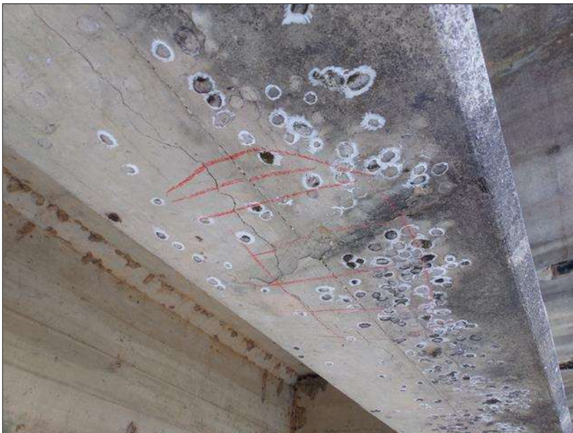
Span 8 Beam 5: 1' long x 8" wide area of delamination on bottom of beam 11' from pier 8.
