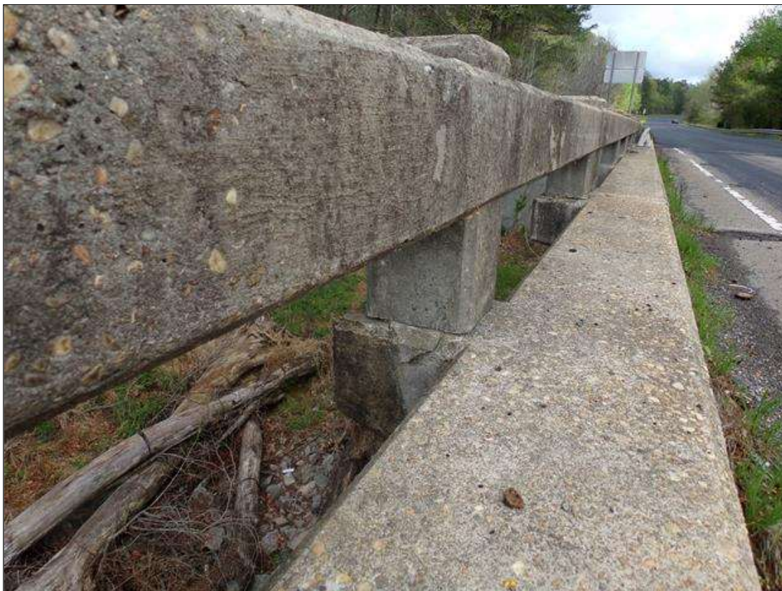
Span 9 Left Bridge Rail: Sound patched area on bottom west face of rail posts 8 and 9.
