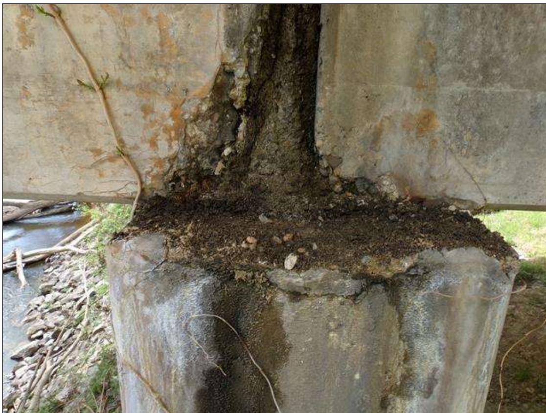
Bent 9 Cap 1: Up to 10" long x full width of top of cap east end area of concrete deterioration with spalling up to 2" deep.
