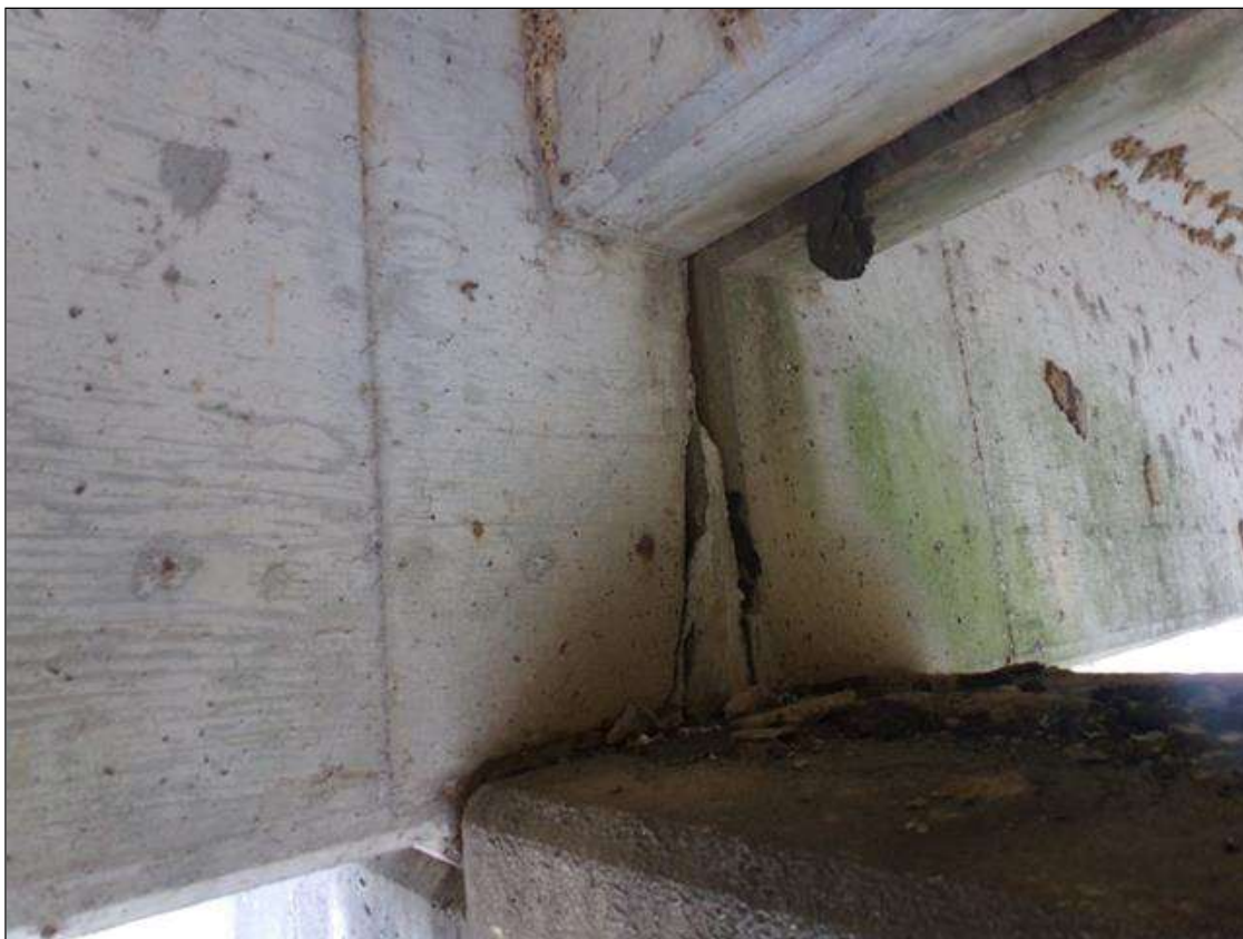
Span 7 Beam 1: End of beam has spalled off 18" high x full width x up to 3" deep over pier 7.
