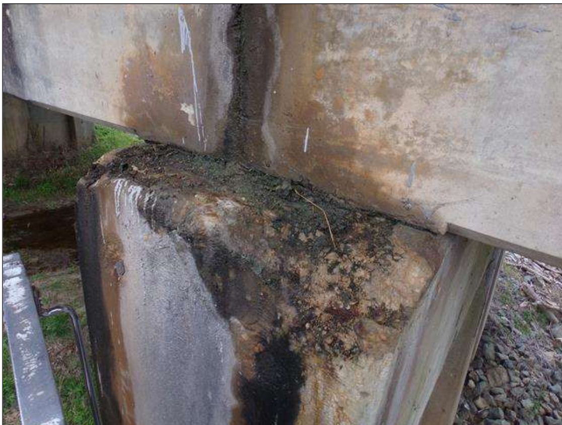
Bent 4 Cap 1: 14" wide x 8" long x 3" deep and 11" wide x 8" long x 2" deep corner spalls on top of cap east end both corners.
