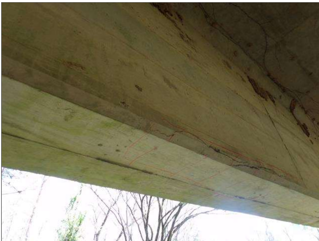
Span 10 Beam 5: Delamination 4' long x 10" wide on bottom of beam x 3" high on west face starting 3' from abutment 2.
