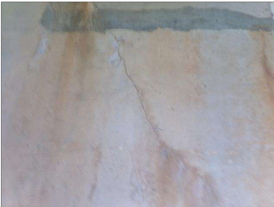
End Bent 1 Abutment/Backwall : 7' long diagonal 1/32" to 1/16" wide crack in front face under beam 2 starting at top of abutment..
