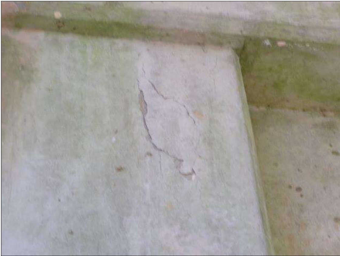
Bent 4 Pile 2: 18" wide x 1' high area of delamination on south face of column starting at bottom of cap.
