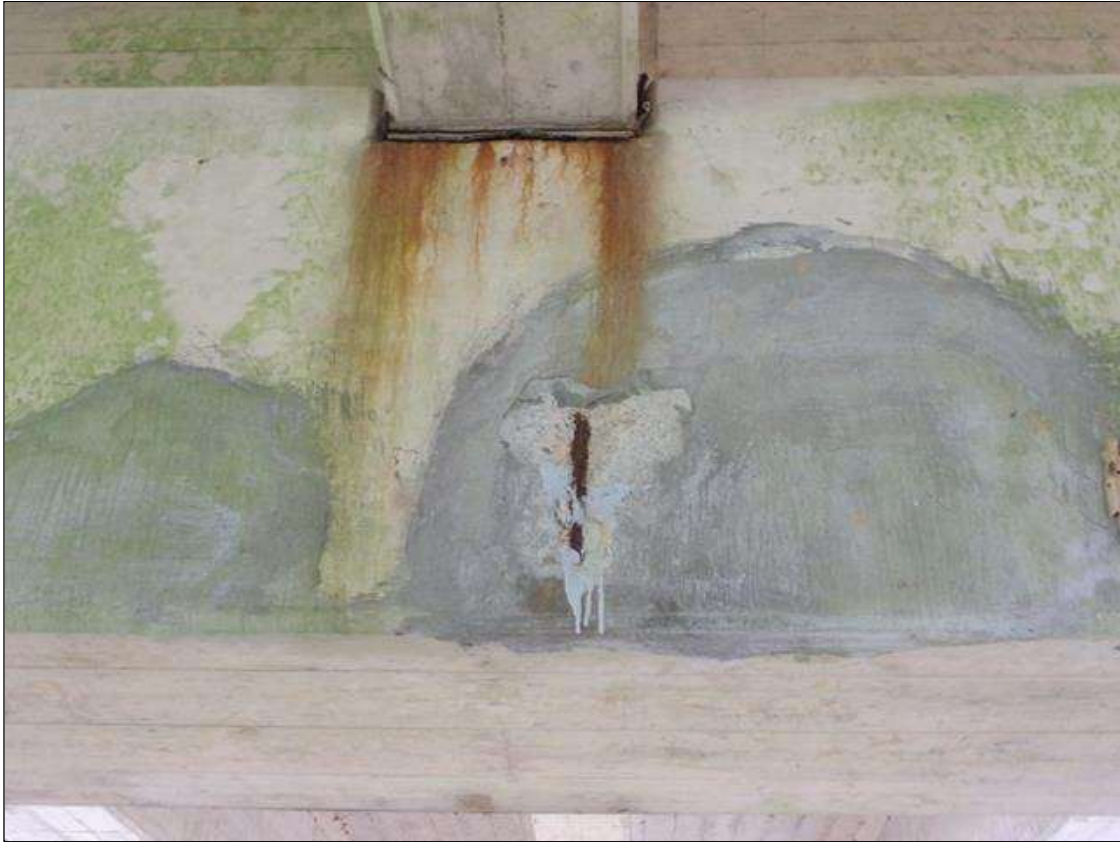
Bent 1 Cap 1: 1' high x 10" wide x 3/4" deep spall with exposed rebar with no measurable section loss on south face of cap under beam 3.
