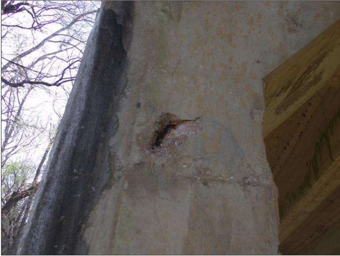
Bent 3 Pile 3: 6" diameter spall 1" deep with exposed rebar with no measurable section loss on north face of column 7' from ground.
