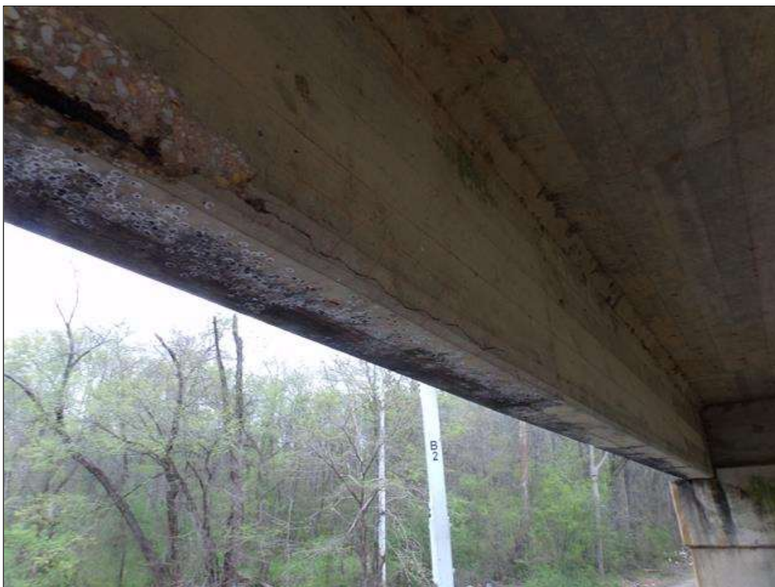
Span 6 Beam 5: Area of delamination 6' long x up to 1' high on west face x up to 10" wide on bottom of beam 16' from pier 6
