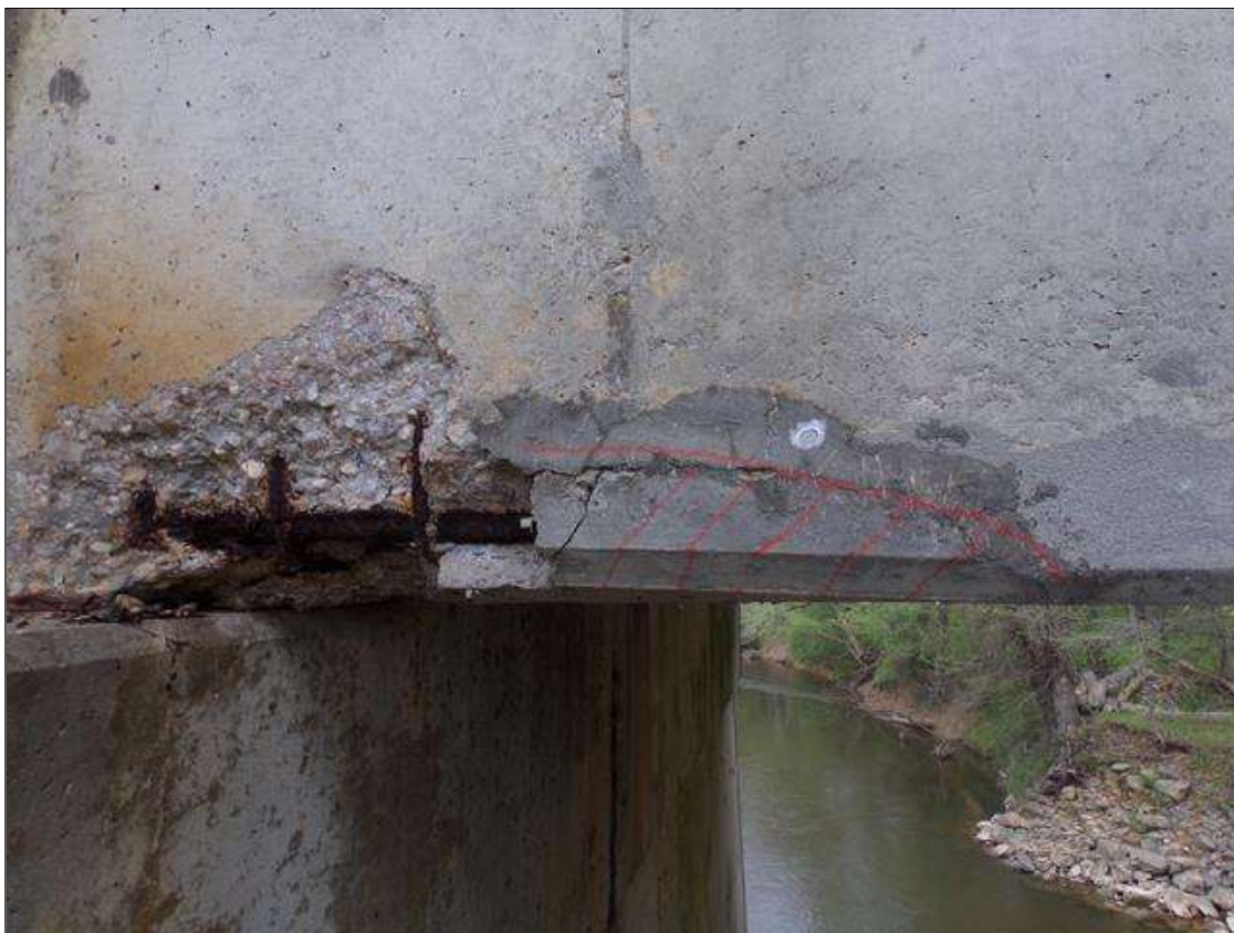
Span 5 Beam 1: Spall 18" long x 1' high on west face x 10" wide on bottom of beam with exposed rebar with no measurable section loss and an area of delamination 16" long x 5" high x 5" wide starting at pier 5.
