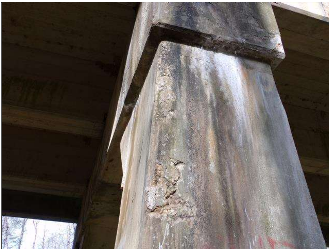
Bent 3 Pile 3: 1' square area of concrete deterioration with spalling up to 1/2" deep 7' from ground line on east face.
