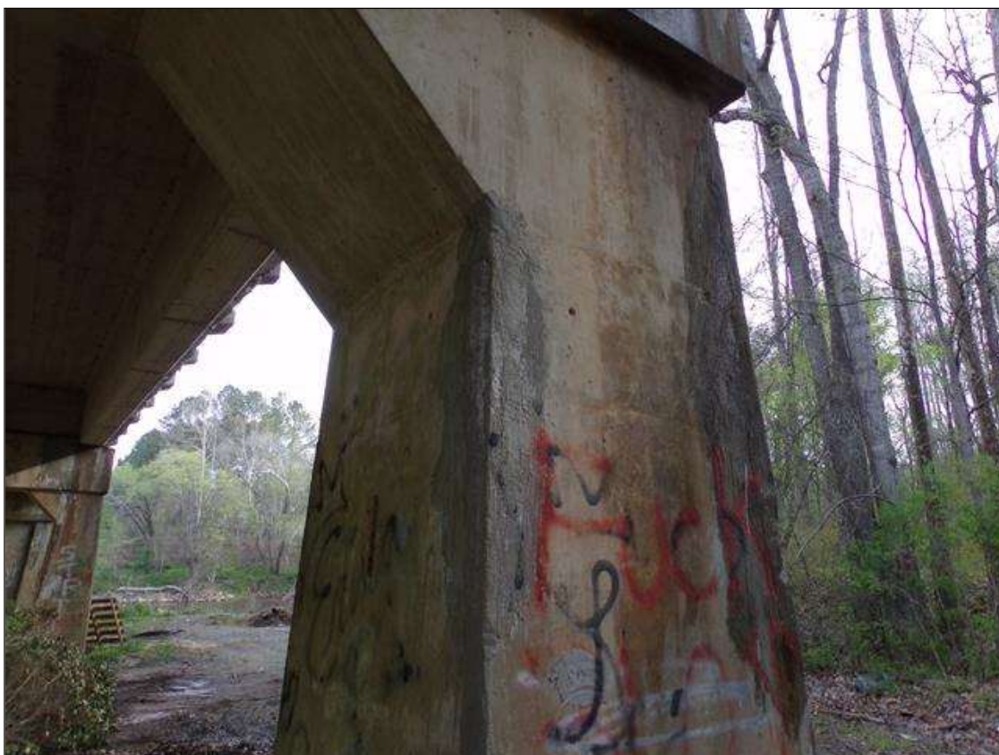
Bent 2 Pile 3: 2.5' high x 7" wide sound corner patch on southwest corner starting 2' from bottom of cap
