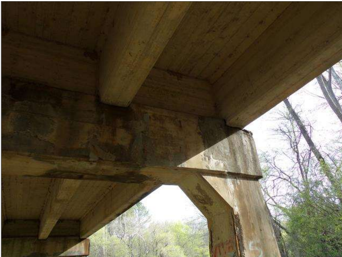
Bent 3 Cap 1: Several sound patched areas on south face of cap starting under bay 2 out to east end.
