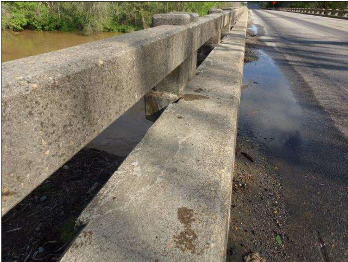
Span 4 Left Bridge Rail: Sound patched area on west face of curb between rail posts 5 and 6 and rail posts 7 and 8.
