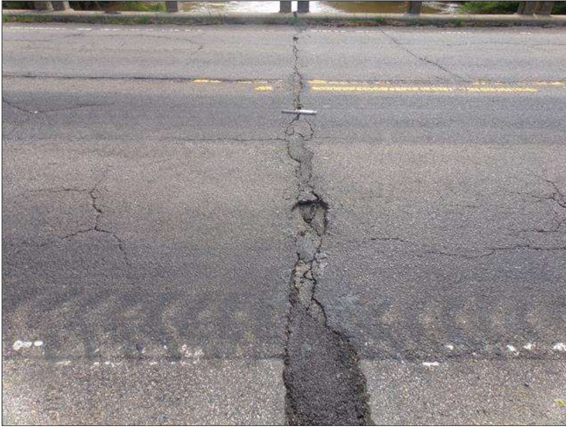
Span 8 Deck: Full width transverse cracks up to 2" wide with areas of potholes up to 3" long x 5" wide x 1" deep over pier 7.
