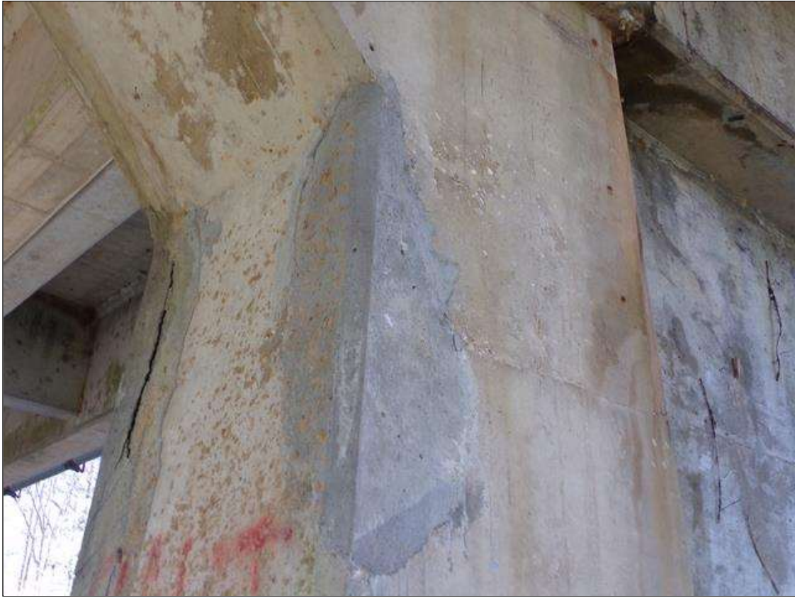
Bent 3 Pile 2: 3' high x 8" wide corner patch on northeast corner that is sound starting 2' from bottom of cap.
