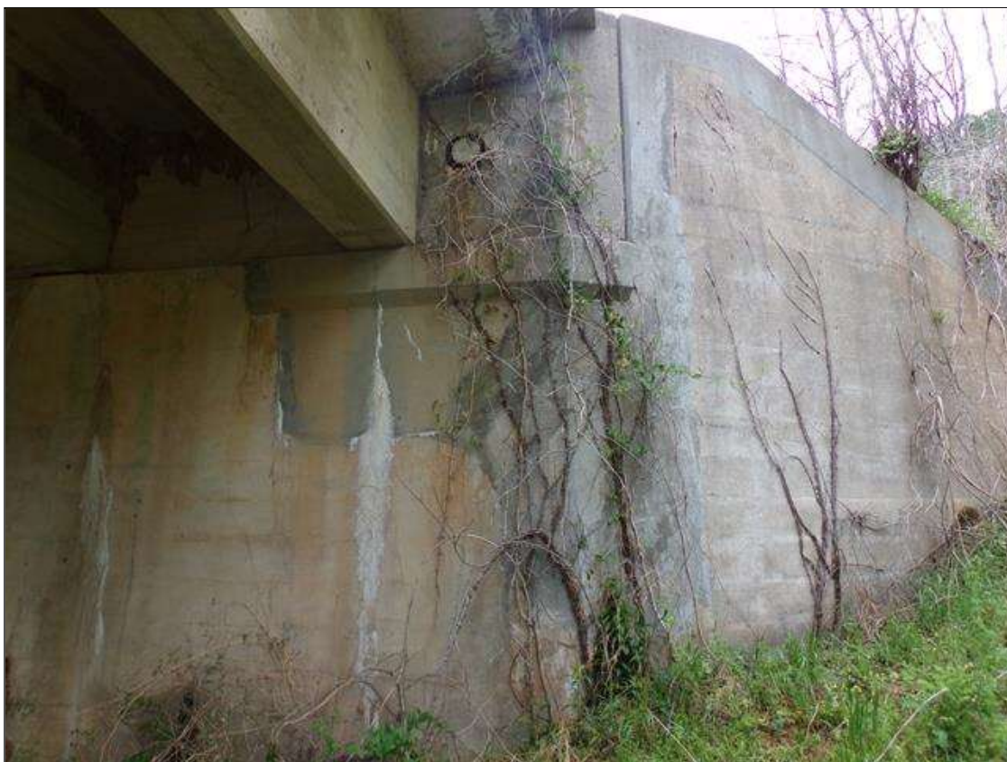
End Bent 2 Abutment/Backwall : 4' high x up to full height sound patched area starting under beam 5 that extends out to east side of beam 5.
