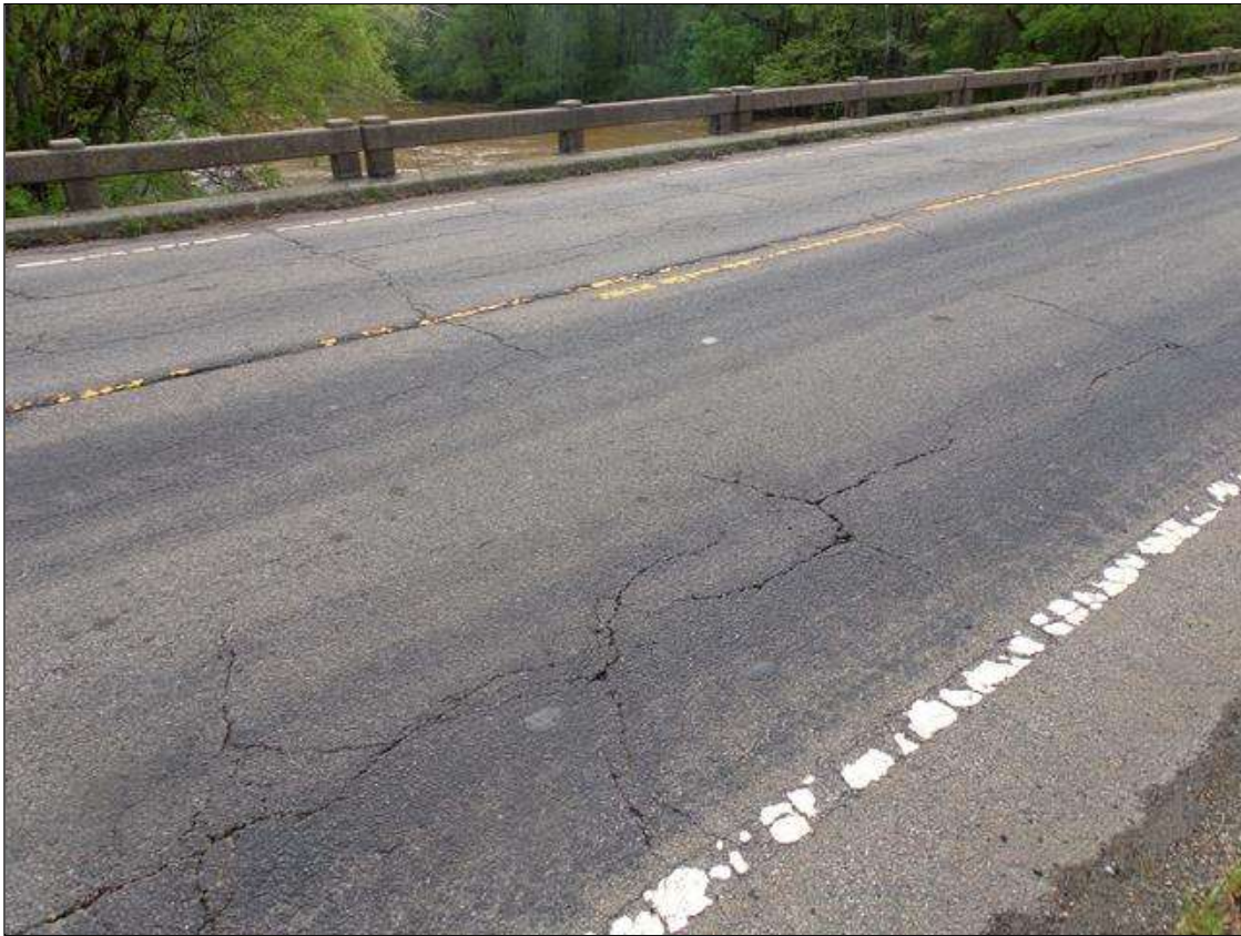
Typical transverse/longitudinal/map cracking in AWS up to 1/2" wide throughout span both travel lanes, span 9 shown
