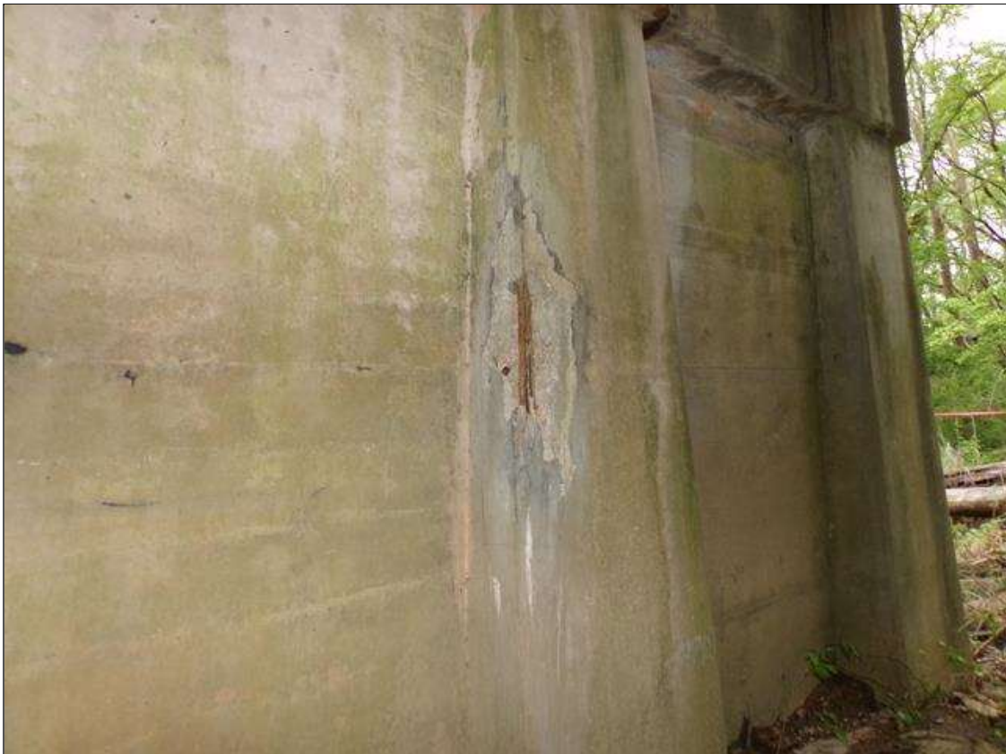
Bent 9 Pile 2: Spall 2' high x 1' wide x 2" deep with exposed rebar with no measurable section loss on north face of column starting 5' from ground line.
