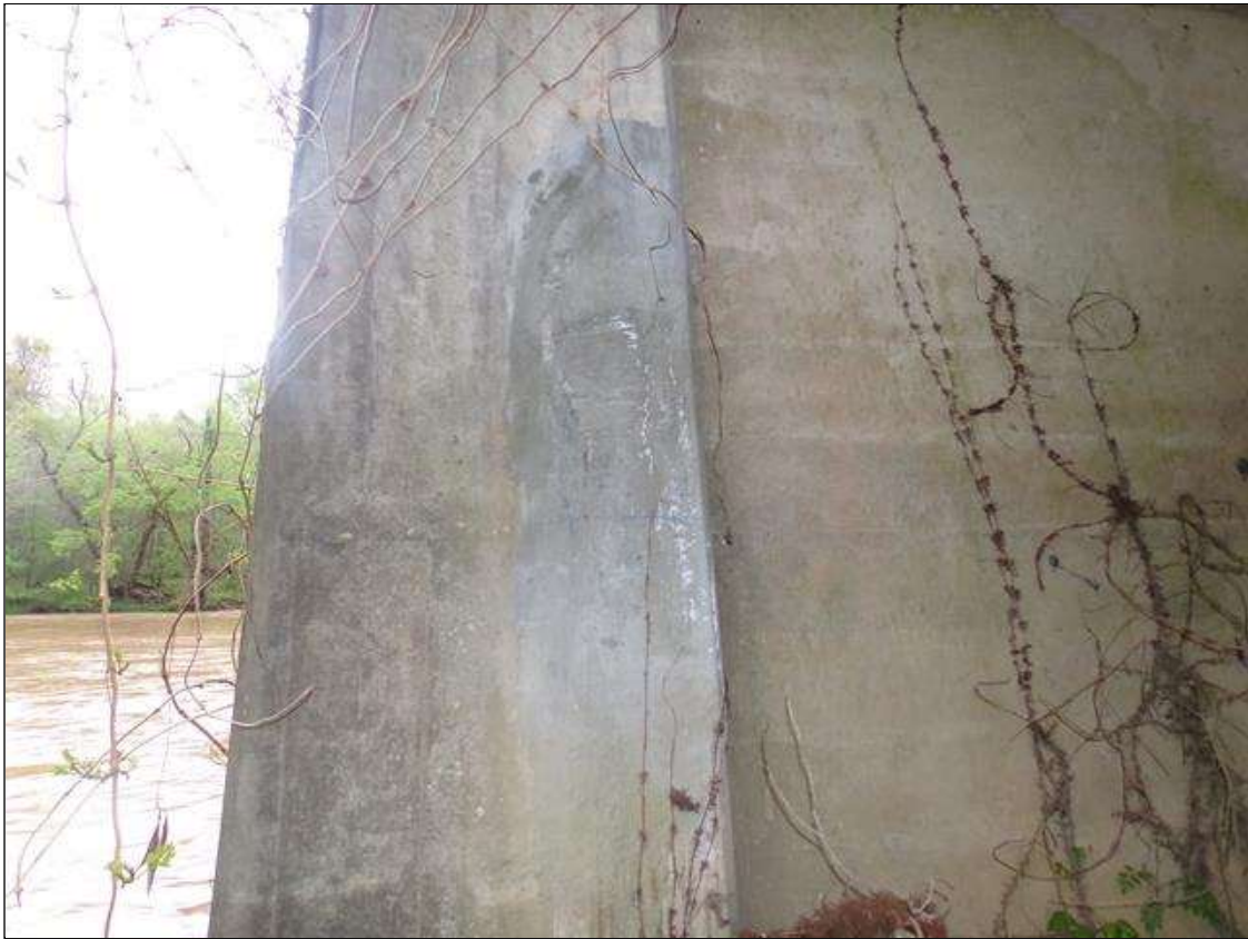
Bent 9 Pile 3: Unsound patched area on north face of column 5' high x 1.5' wide with a 1/32" x 2' long crack at top of patch starting at bottom of cap.
