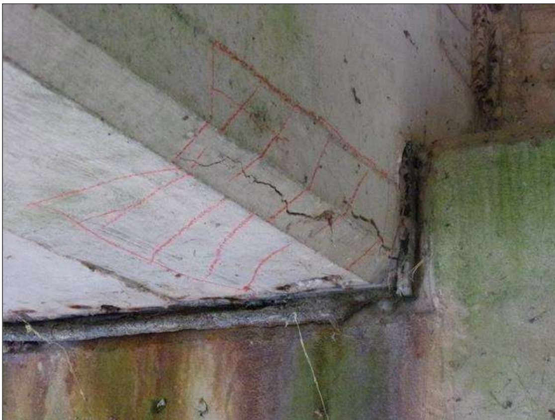
Span 5 Beam 4: 1" long x 4" high on west face x 6" wide on bottom of beam delamination with a crack up to 1/8" wide full width of delamination starting at pier 4.
