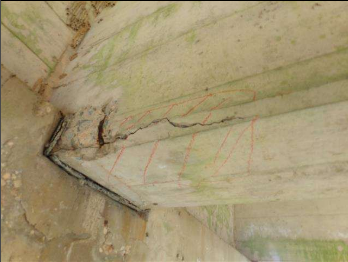
Span 4 Beam 4: Area of delamination 21" long x 3" high on west face x 10" wide on bottom of beam with a 10" wide x 8" high x 2" deep spall with exposed rebar with no measurable section loss at pier 4.
