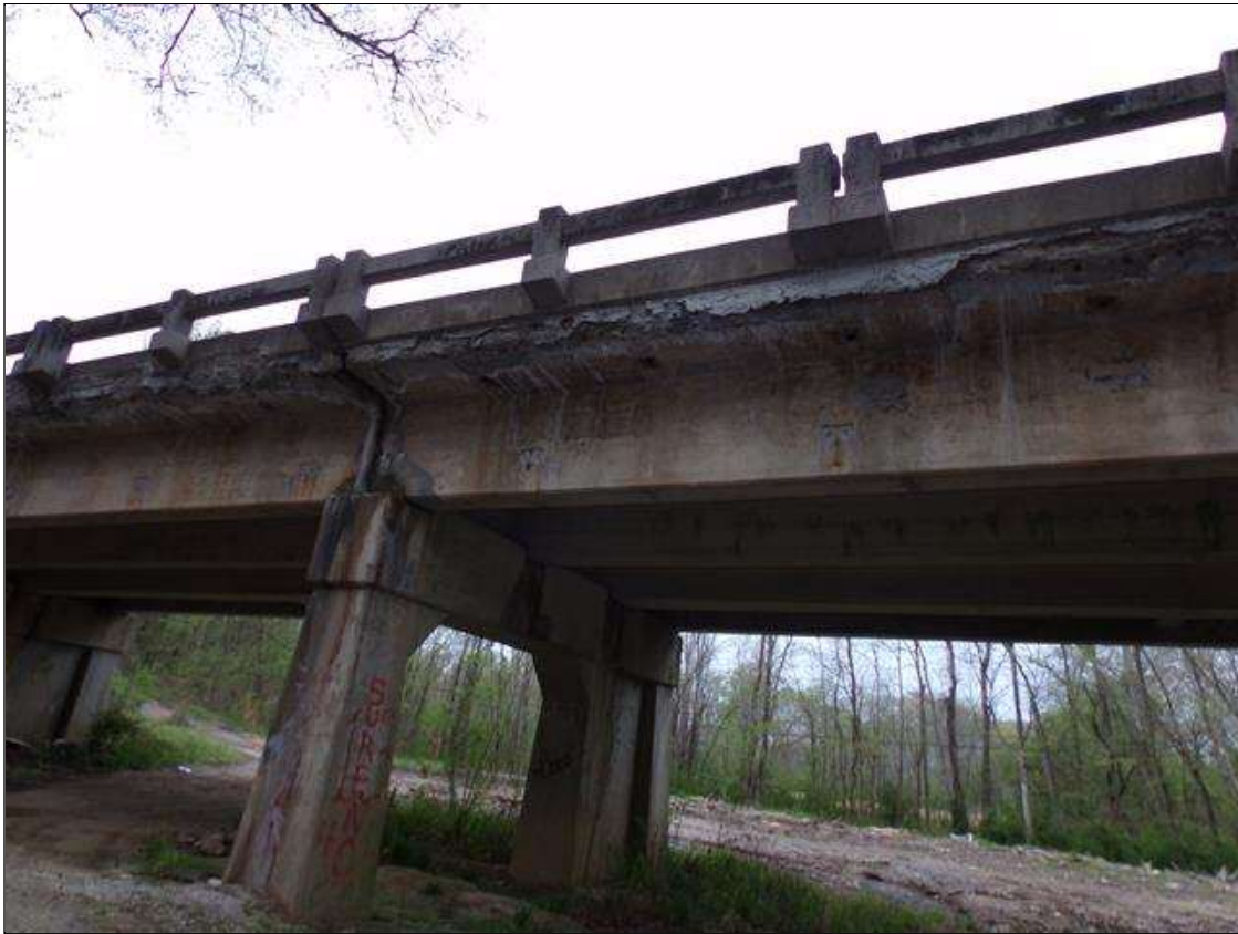
Span 3 Deck: Patched area 1' high x full length of east overhang that is distressed with efflorescence/stalactites/staining and cracking throughout
