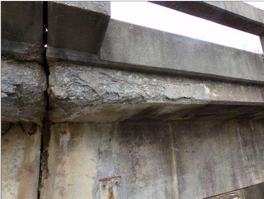
Span 7 Deck: 6' long x full height of front face east overhang area of concrete deterioration with a spall 2' long x 7" wide x up to 2" deep starting at pier 6.
