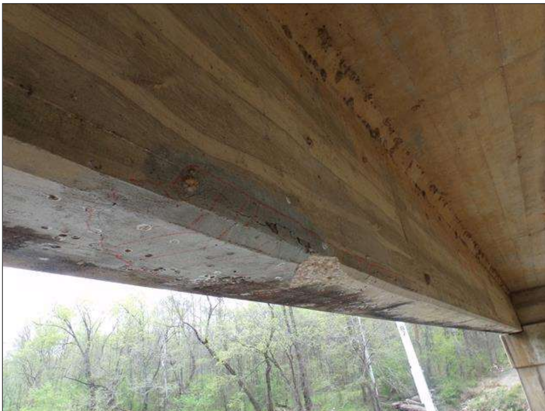
Span 7 Beam 5: Delamination 8' long x up to full width on bottom of beam x 4" high on west face with a 10" diameter spall x 2" deep on bottom of beam starting 3' from pier 7.
