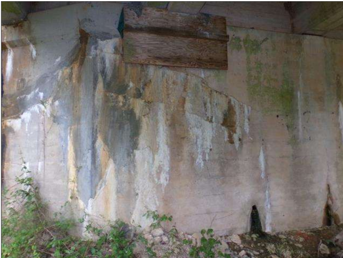
End Bent 2 Abutment/Backwall : Two 6' long x up to 1/32" wide horizontal cracks with efflorescence and a 6' high x 4' wide sound patched area under beams 2 and 3.
