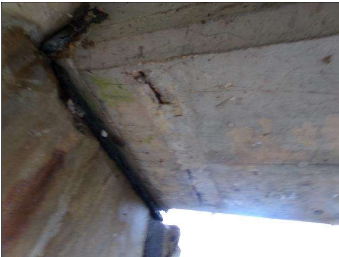
Span 5 Beam 5: Spall 1" wide x full width of bottom of beam x 1/4" deep at pier 5.
