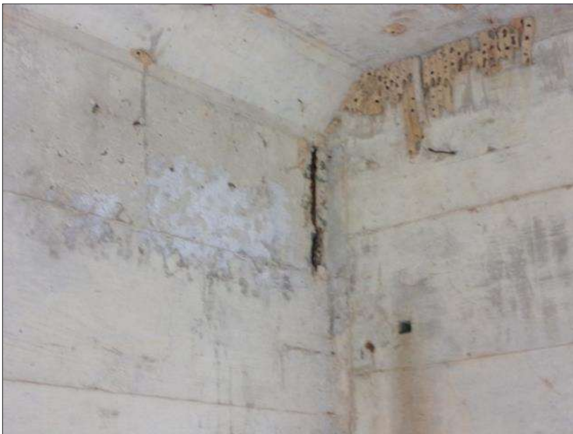
Span 3 Beam 5: 1' high x 3" wide x 1" deep spall with exposed rebar with no measurable section loss on west face of beam over pier 2.
