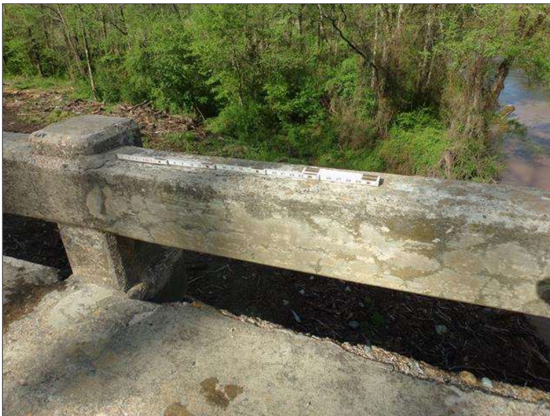
Span 4 Left Bridge Rail: 2' long x 1/8" wide crack in top of top rail at rail post 8.
