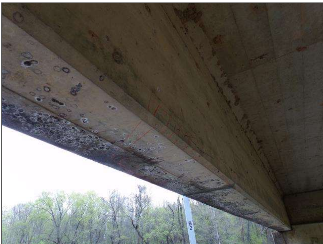
Span 8 Beam 5: Delamination 4' long x up to 11" wide on bottom of beam x 4" high on west face 20' from pier 8.
