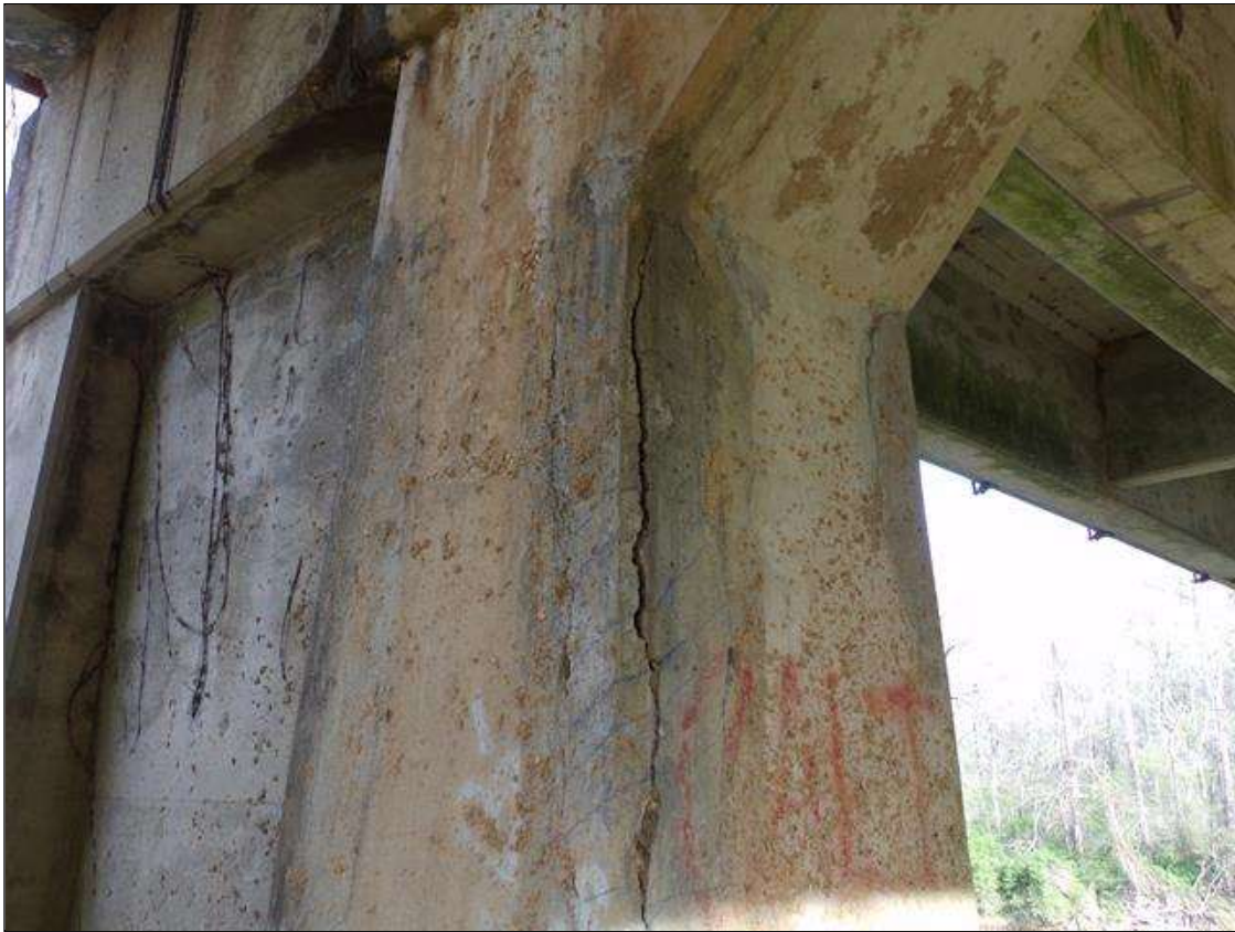
Bent 3 Pile 2: 5' high x 8" wide corner patch on southeast corner that is unsound with a crack up to 1/8" wide that extends down to ground starting 2' from bottom of cap.
