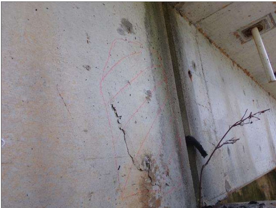
Span 9 Beam 1: 2' square area of delamination on west face of beam over pier 8.
