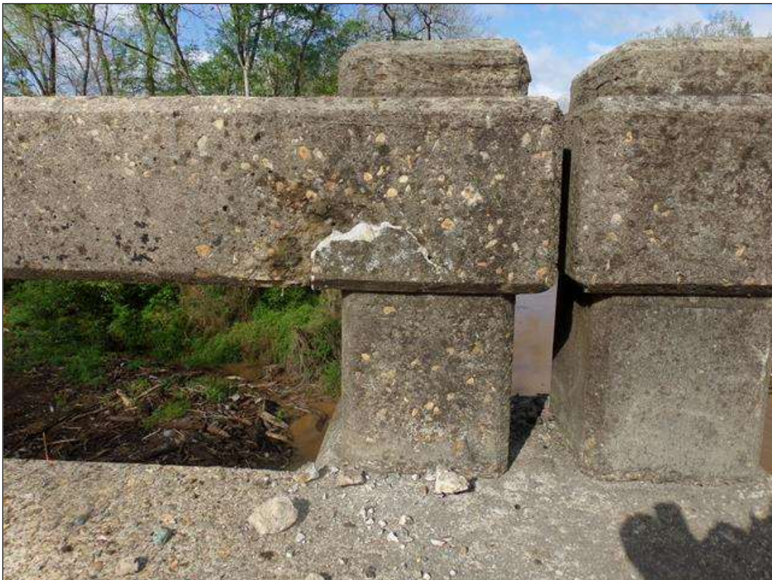
Span 5 Left Bridge Rail: Full height up to 1/16" crack with a 8" long x 4" high area of delamination/spall up to 3/4" deep in front face of post.
