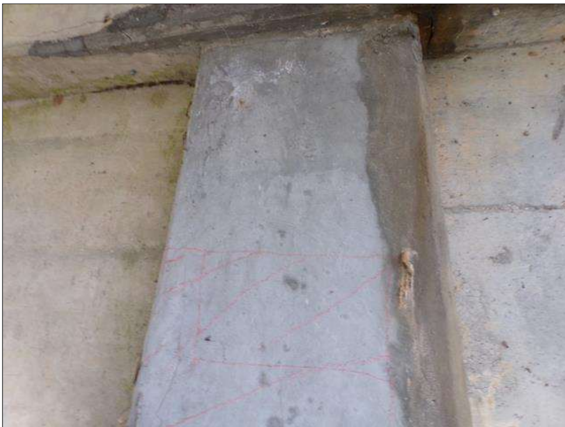
Bent 4 Pile 2: 3' square sound patched area with a 1/32" vertical crack north face starting at bottom of cap
