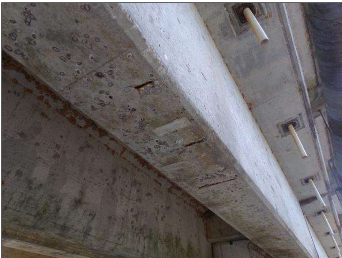
Span 8 Beam 1: Three spalls spaced 1' apart up to 10" long x 1" wide x 1/4" deep with exposed rebar with no measurable section loss on bottom of beam 14' from pier 7
