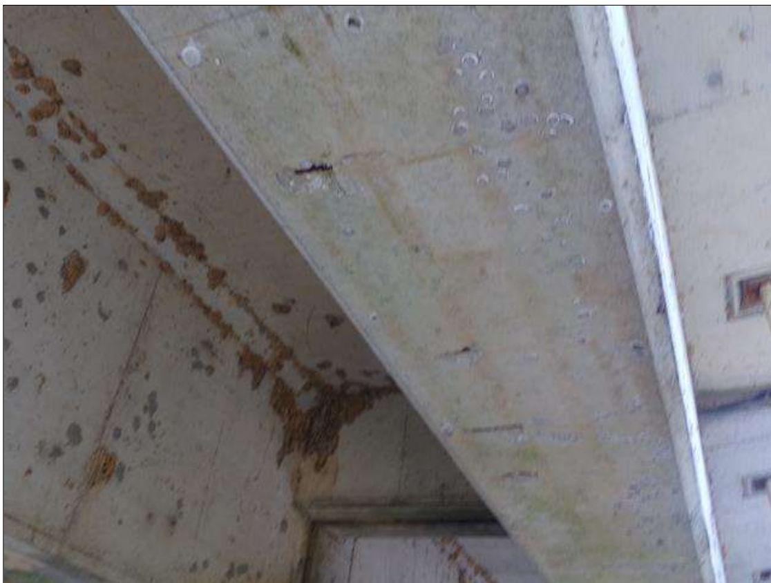
Span 9 Beam 1: 4 spalls spaced approximately 1' apart up to 3" long x 2" wide x 1/2" deep with exposed rebar with no measurable section loss on bottom of beam 7' from pier 8.
