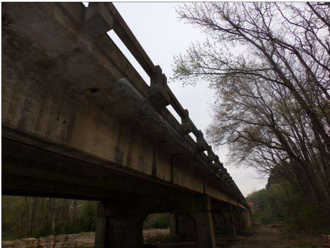
Span 1 Deck: Patched area 1' high x full length of east overhang that is distressed with efflorescence/stalactites/staining and cracking throughout .
