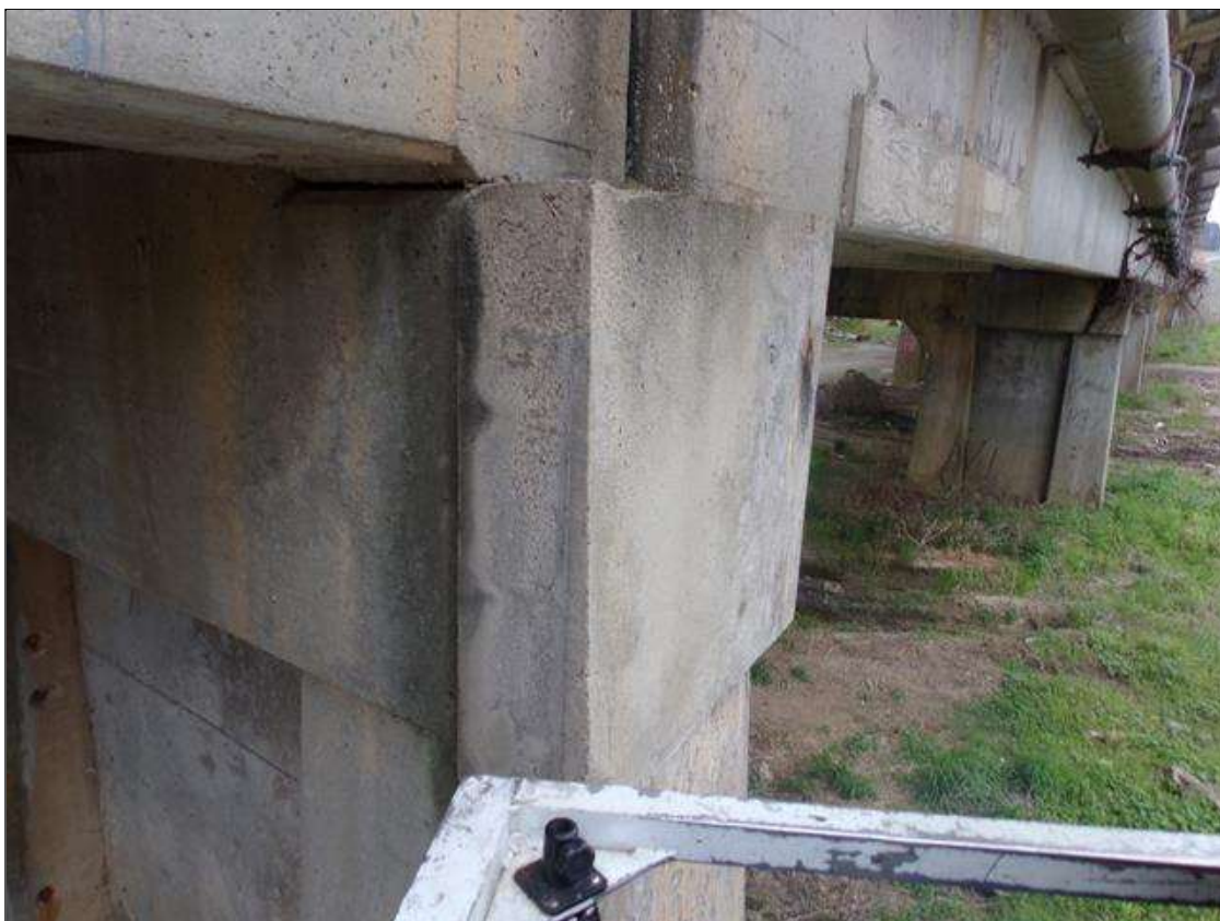
Bent 4 Cap 1: 6" deep x full height/width sound patched area on west end of cap.
