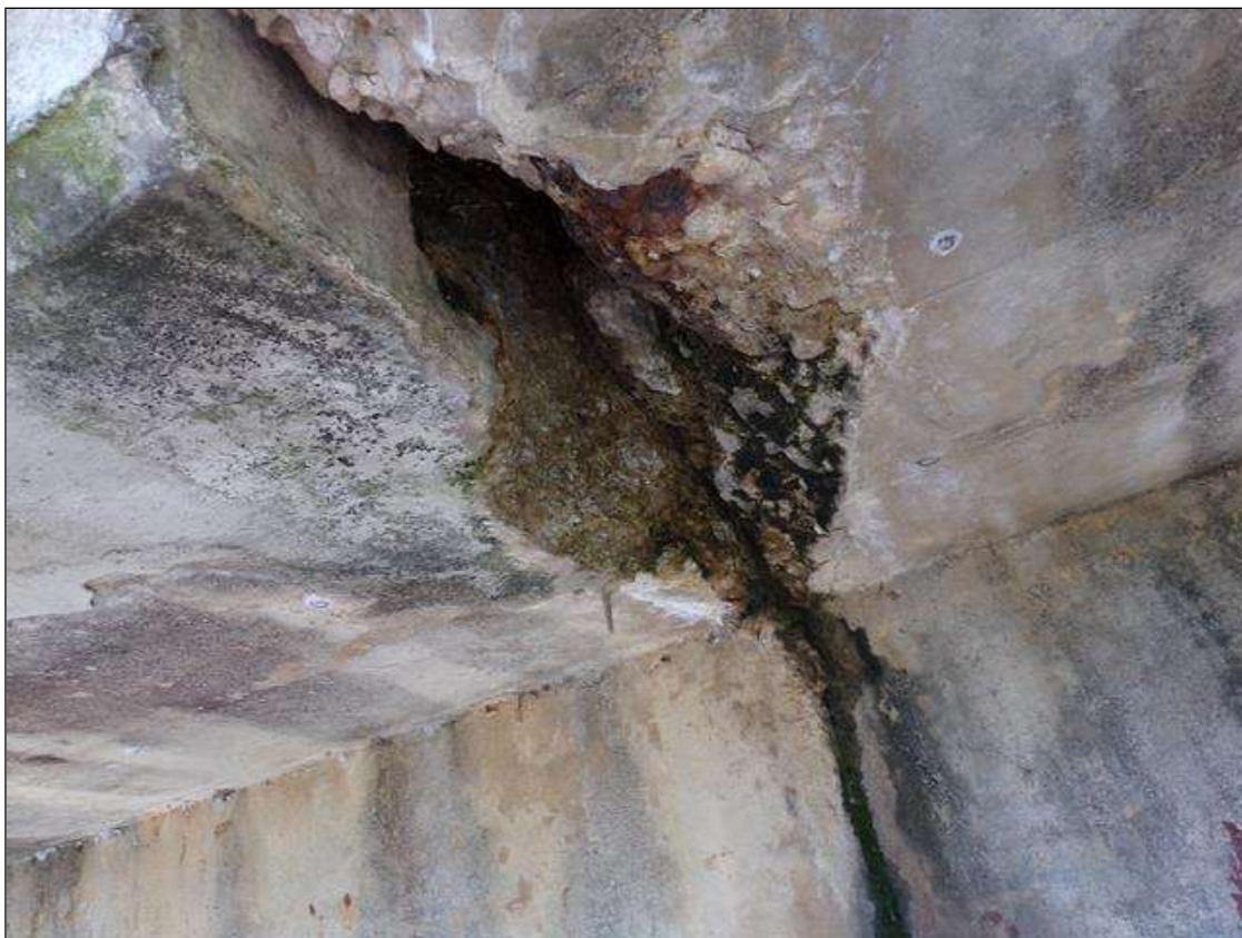
Span 8 Deck: Spall in east overhang 2' wide x 4" long x 5" deep at end of span over pier 8.
