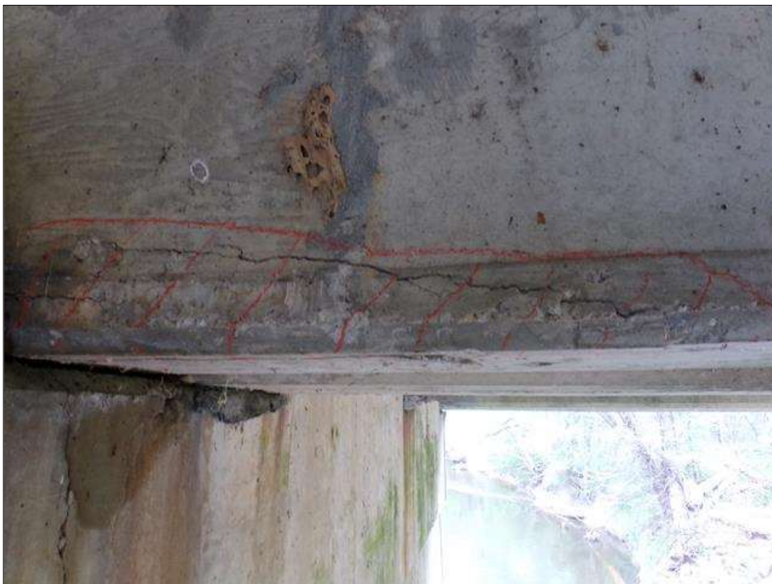
Span 5 Beam 2: 30" long x 10" wide on bottom of beam x 6" high on west face area of delamination starting at pier 5
