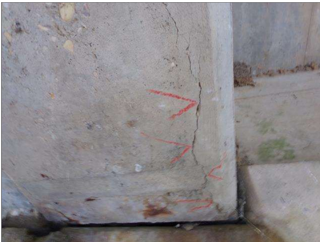
Span 6 Beam 3: 2' long crack 1/16" wide on bottom of beam starting at pier 6.
