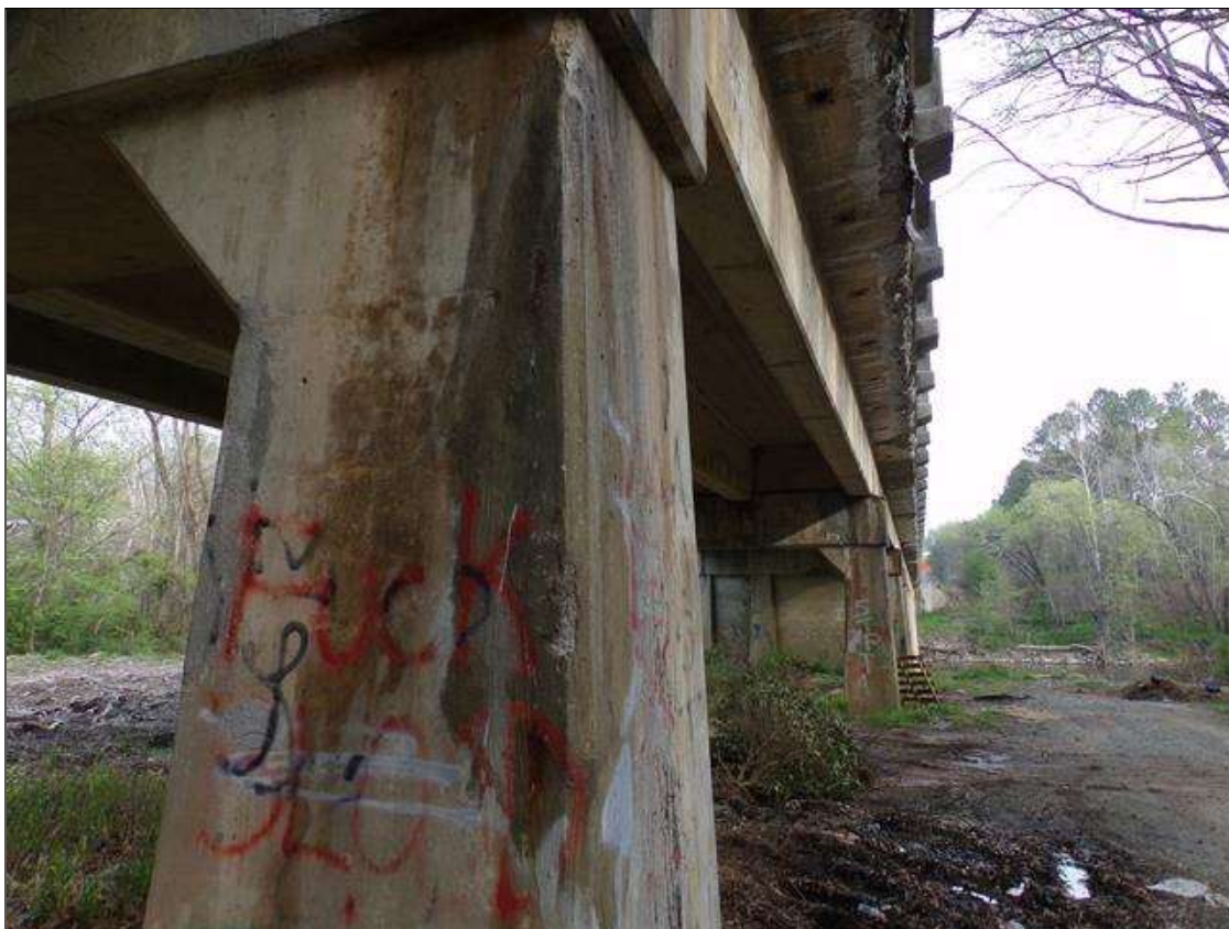
Bent 2 Pile 3: 5' high x 8" wide corner patch on southeast corner that is unsound starting at bottom of cap.
