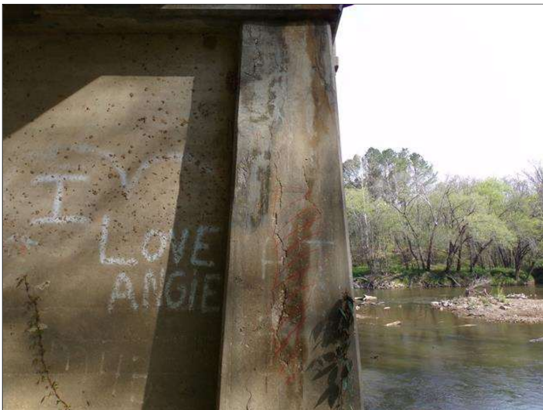
Bent 4 Pile 3: 9' high x 16" wide area of delamination on south face of column starting 3' from ground.
