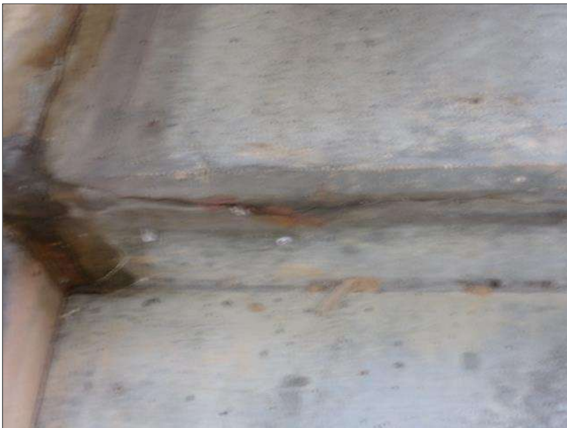
Bent 4 Cap 1: 3' long x 1/8" wide horizontal crack on bottom of cap between columns 1 and 2 starting at construction joint north side.
