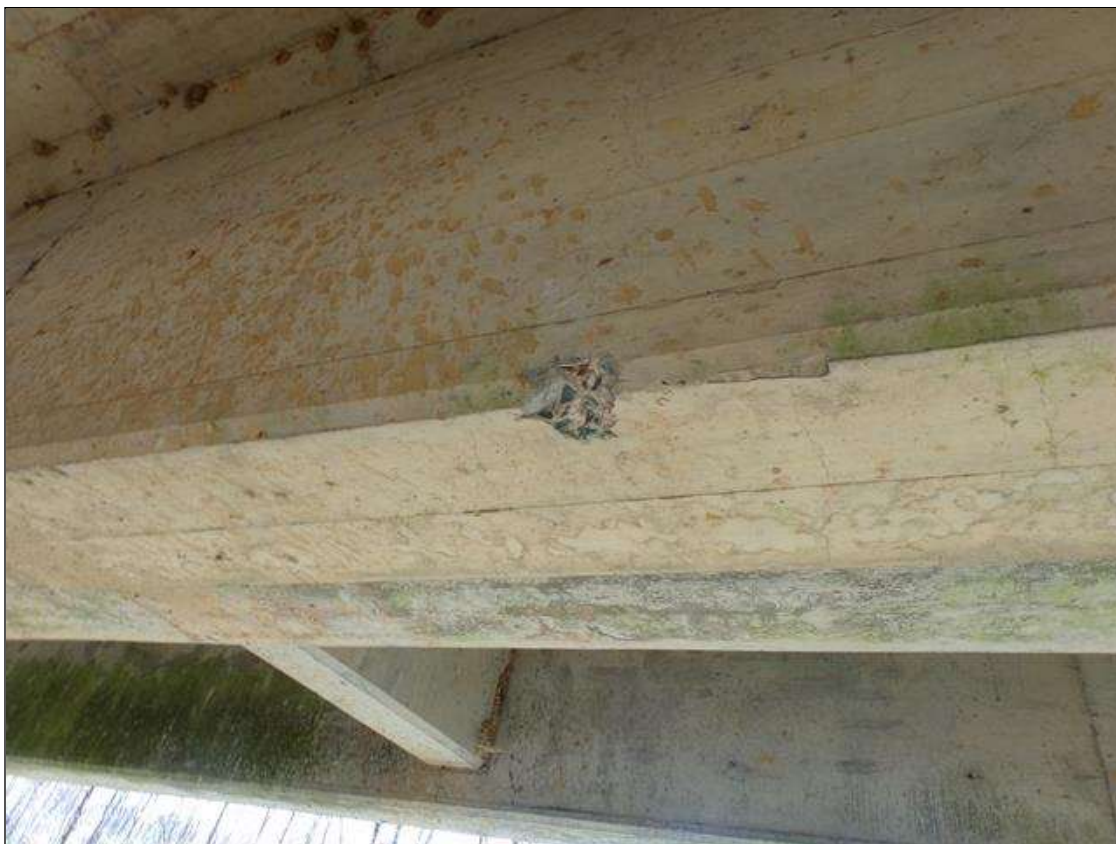
Span 4 Beam 3: 4" diameter corner spall on bottom and east faces 1/2" deep 20' from pier 4.
