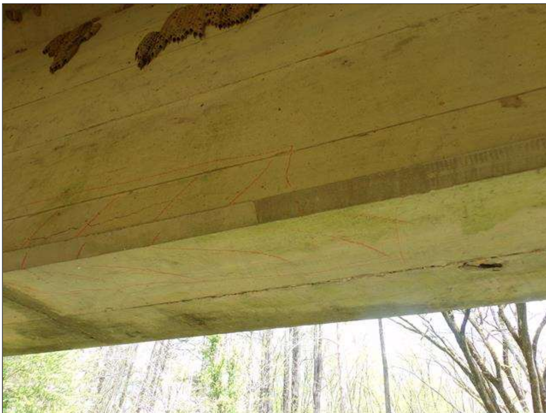
Span 10 Beam 5: Delamination 3' long x 6" wide on bottom of beam x 3" high on west face approximately 14' from pier 9.
