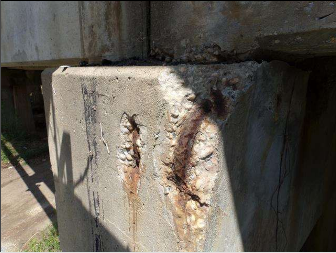
Bent 1 Cap 1: 2 spalls at west end of cap up to 13" high x 8" wide x 2" deep with exposed rebar with no measurable section loss
