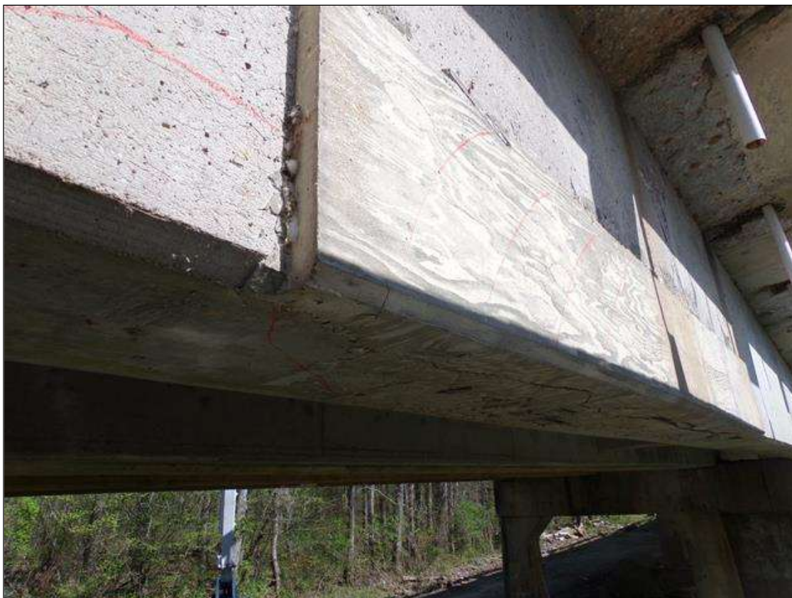
Span 4 Beam 1: Area of delamination 13' long x 15" high on west face x full width of bottom of beam with a 10' long unsound patch starting at pier 4.
