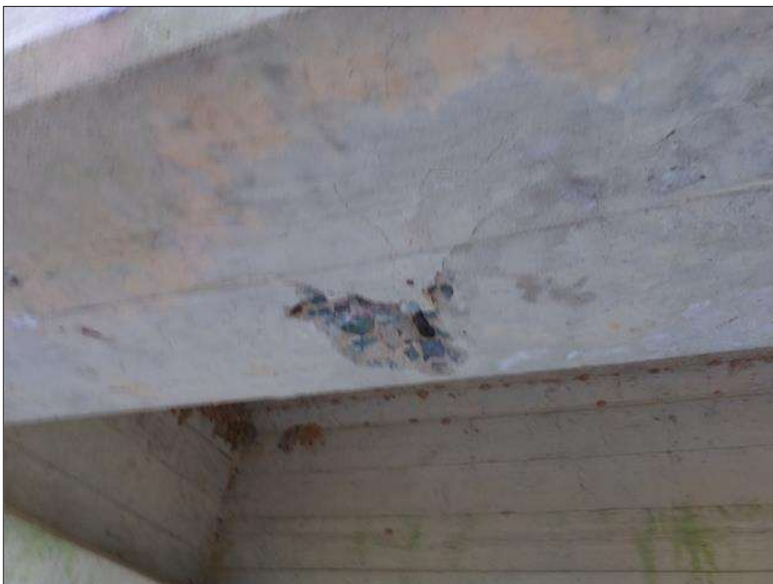
Span 3 Beam 5: 5" diameter spall 1" deep on bottom of beam with exposed rebar with no measurable section loss 5' from pier 2.
