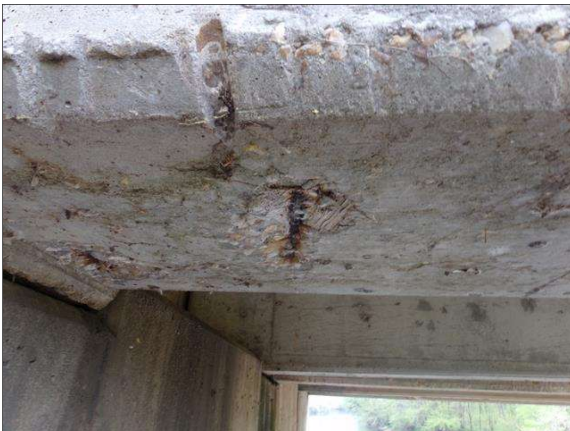
Span 7 Beam 1: 9" long x 6" wide x 1/2" deep spall with exposed rebar with no measurable section loss on bottom of beam 1' from pier 7.
