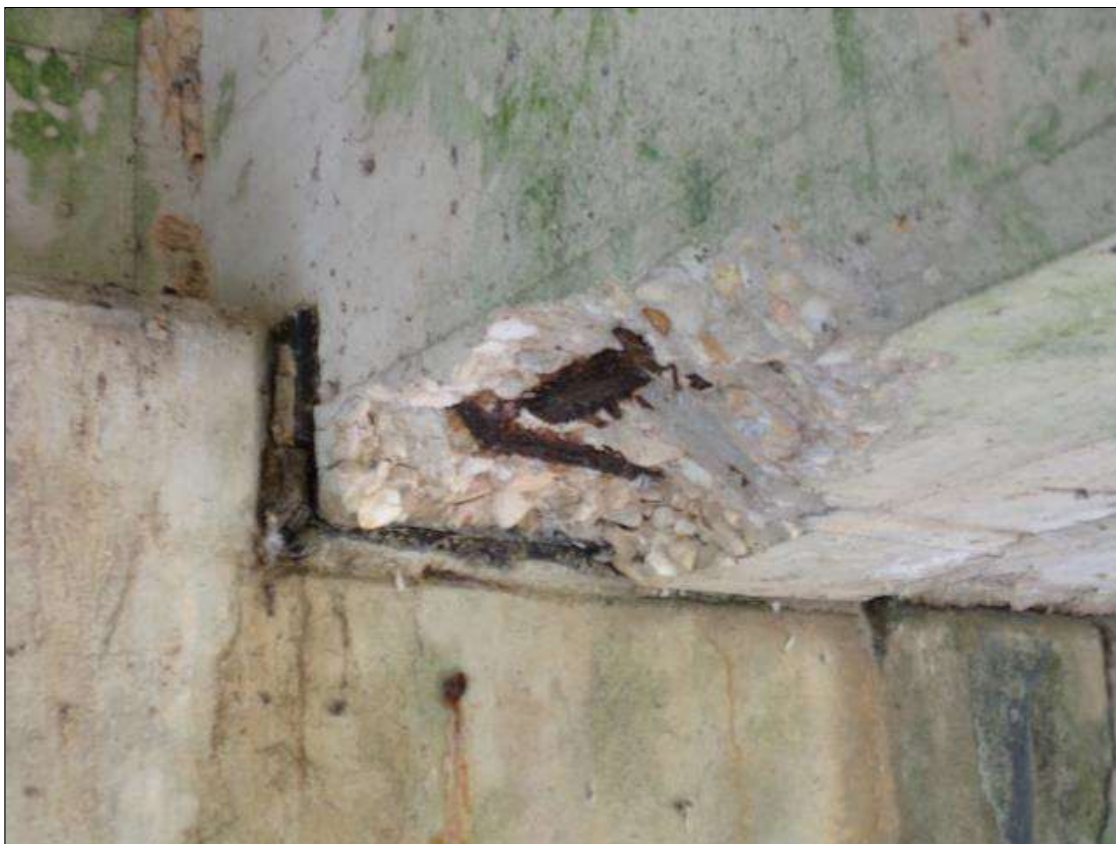
Span 8 Beam 3: Spall 1' square x 3" deep on bottom of beam with exposed rebar with no measurable section loss at pier 7.
