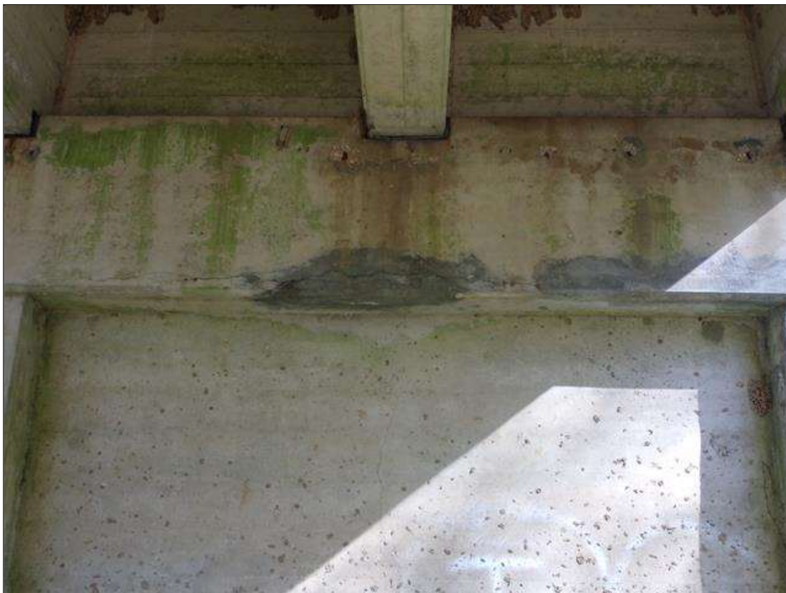
Bent 4 Cap 1: 8' long x 6" wide area of delamination on bottom corner of cap under bays 2 and 3.
