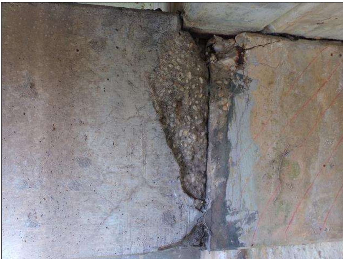
Bent 3 Cap 1: 3' high x up to 16" wide x up to 4" deep spall with exposed rebar with no measurable section loss on south face of cap under beam 2.
