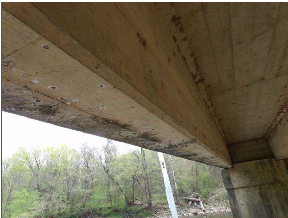
Span 8 Beam 5: Delamination 4' long x 8" wide on bottom of beam x 4" high on west face 13' from pier 8.
