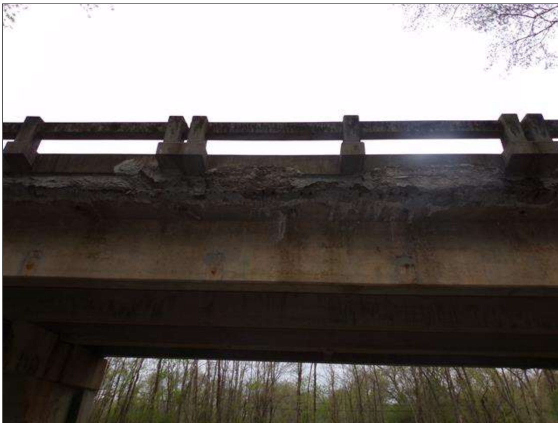
Span 2 Deck: Patched area 1' high x full length of east overhang that is distressed with efflorescence/stalactites/staining and cracking throughout
