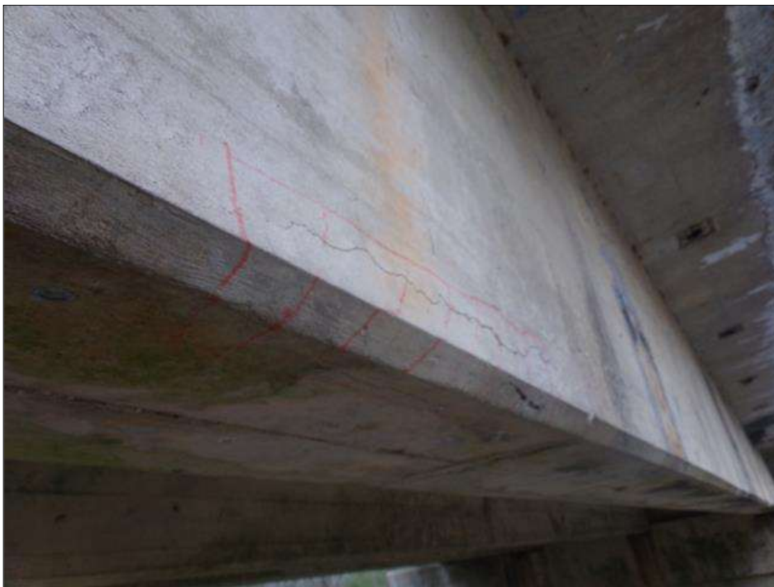
Span 5 Beam 5: 18" long x 3" high on east face x 2" wide on bottom of beam starting 7' from pier 4.
