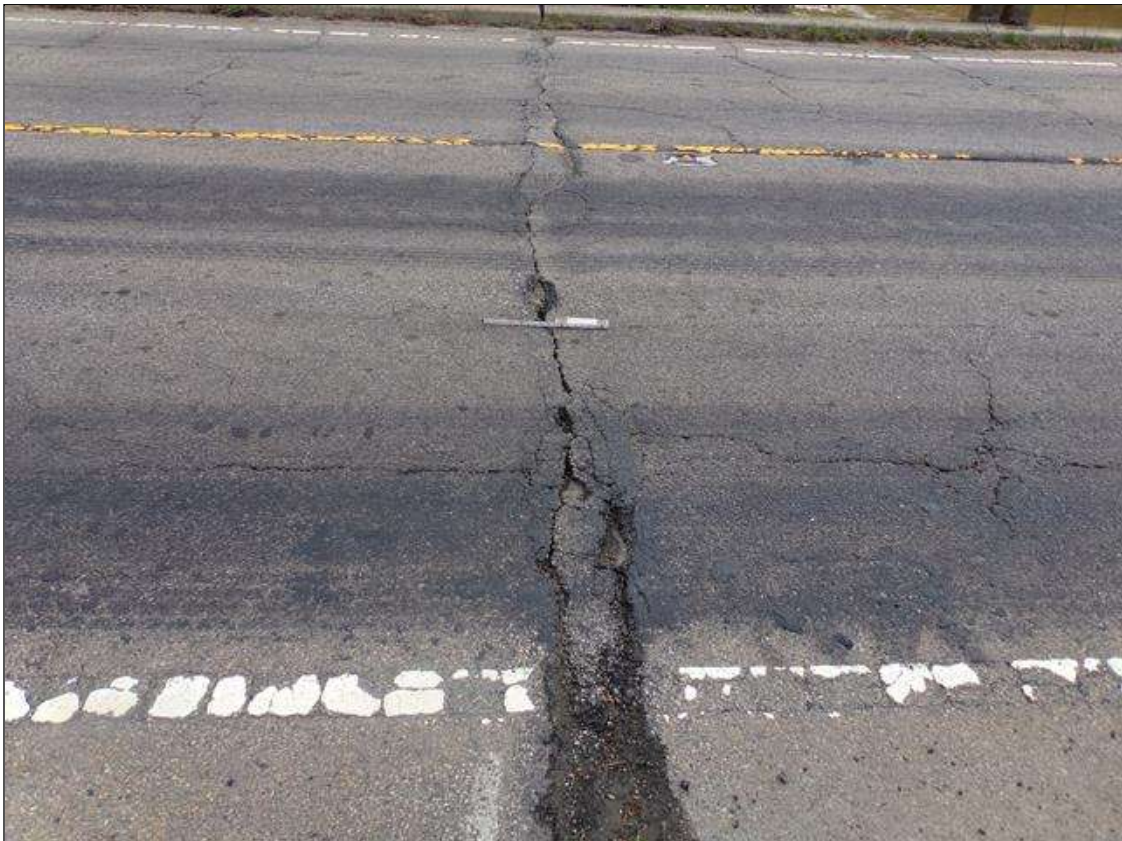
Span 10 Deck: Full width transverse cracks up to 1" wide with areas of potholes up to 6" long x 3" wide over pier 9.
