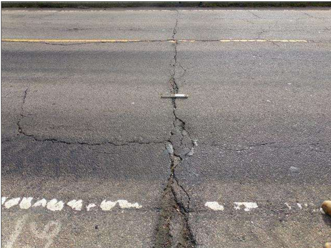
Span 9 Deck: Full width transverse cracks up to 1" wide with areas of potholes up to 1" long x 3" wide x 1/4" deep over pier 8.
