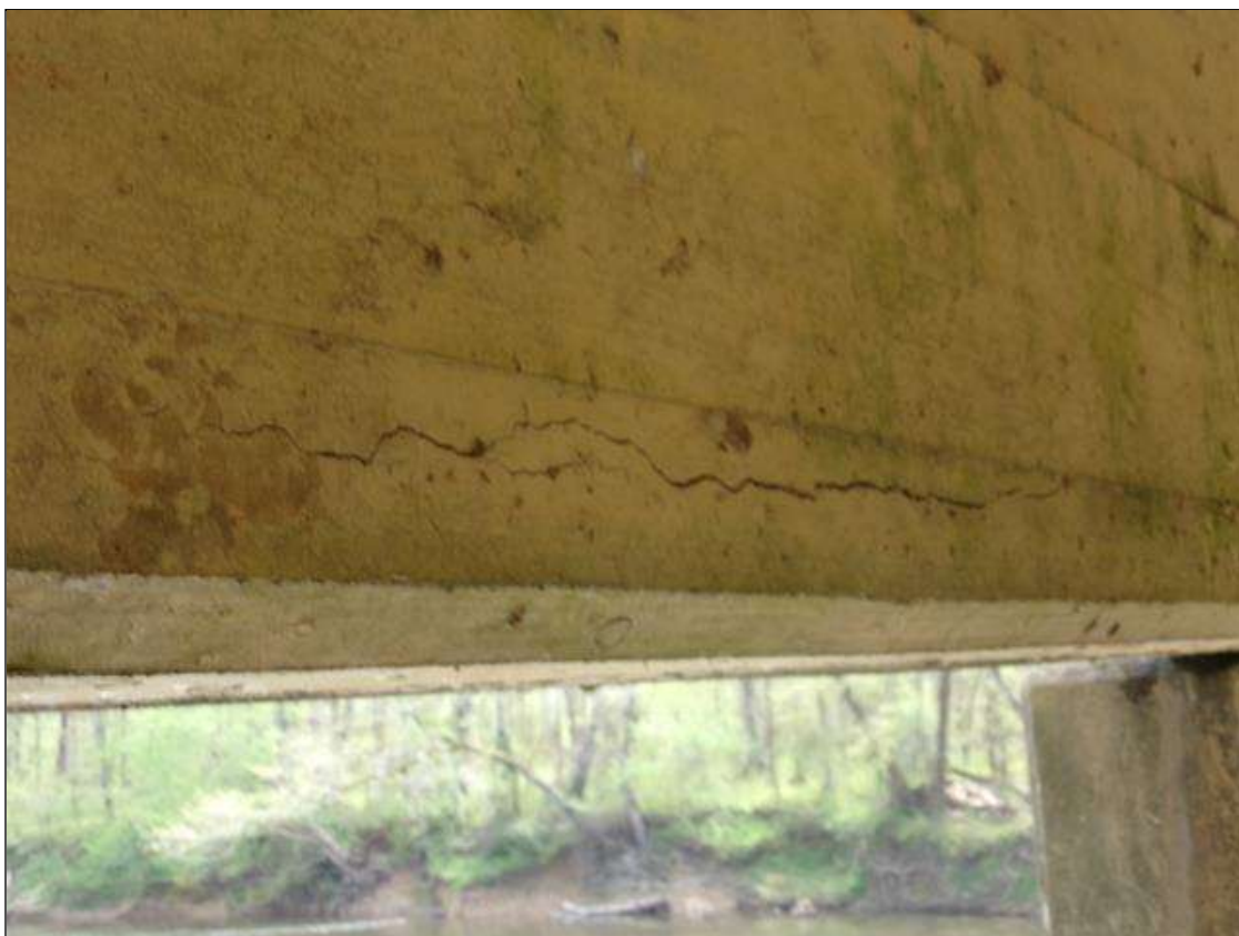
Span 9 Beam 5: 3' long horizontal crack 3/16" wide on west face of beam starting 5' from pier 8
