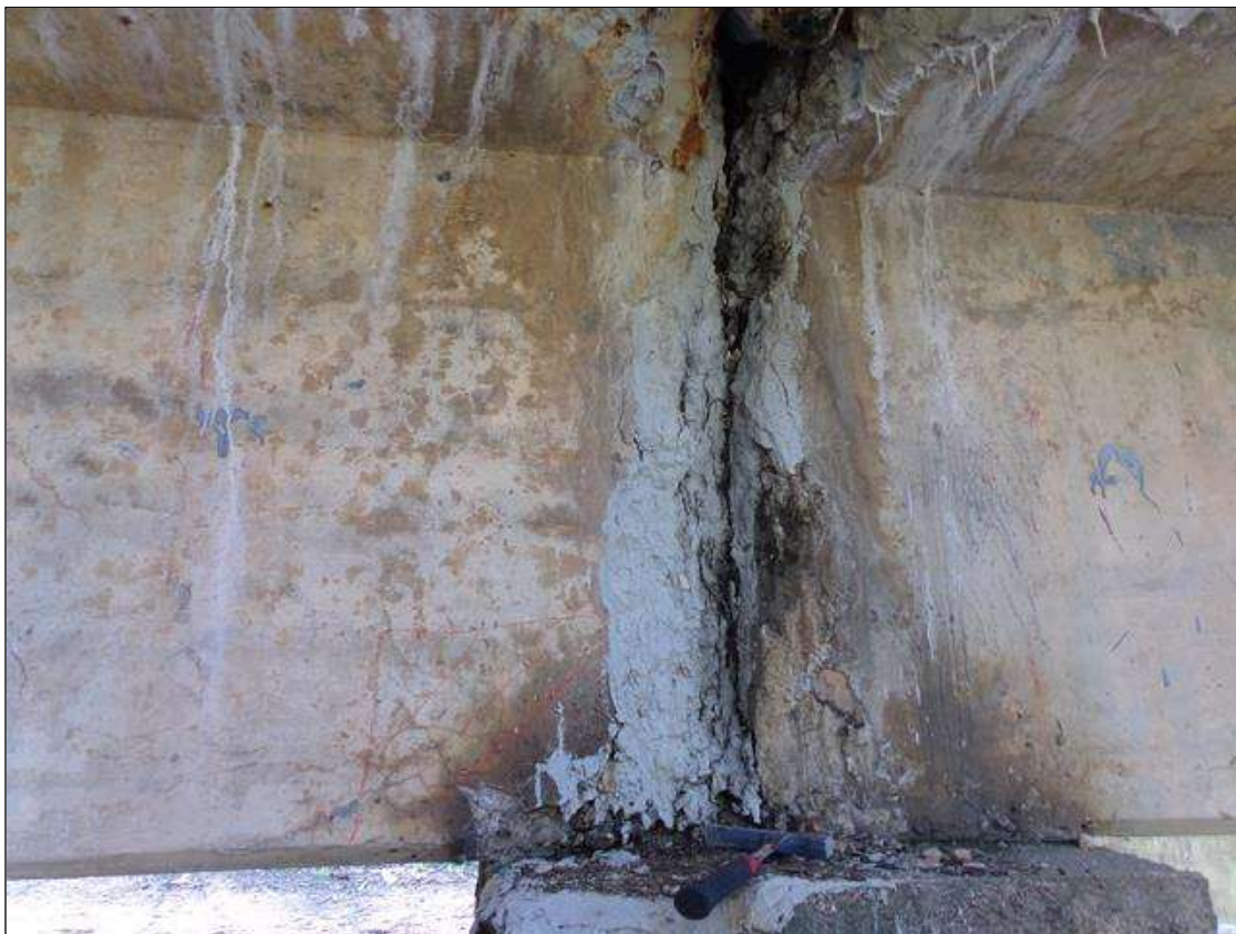
Span 3 Beam 5: 1' square area of delamination on east face of beam at pier 3.
