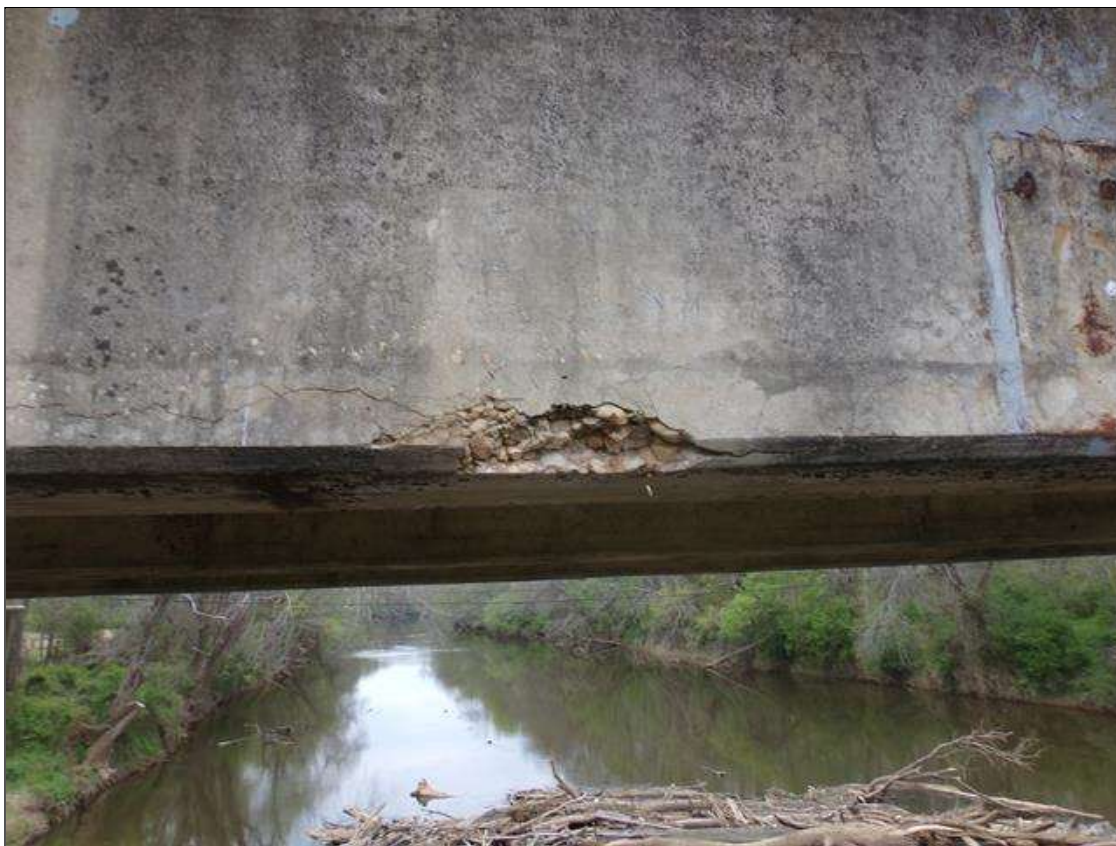
Span 6 Beam 5: 1' long x 4" high x 2" deep spall on east face of beam with cracking up to 3' long x up to 3/16" wide on both sides of spall.
