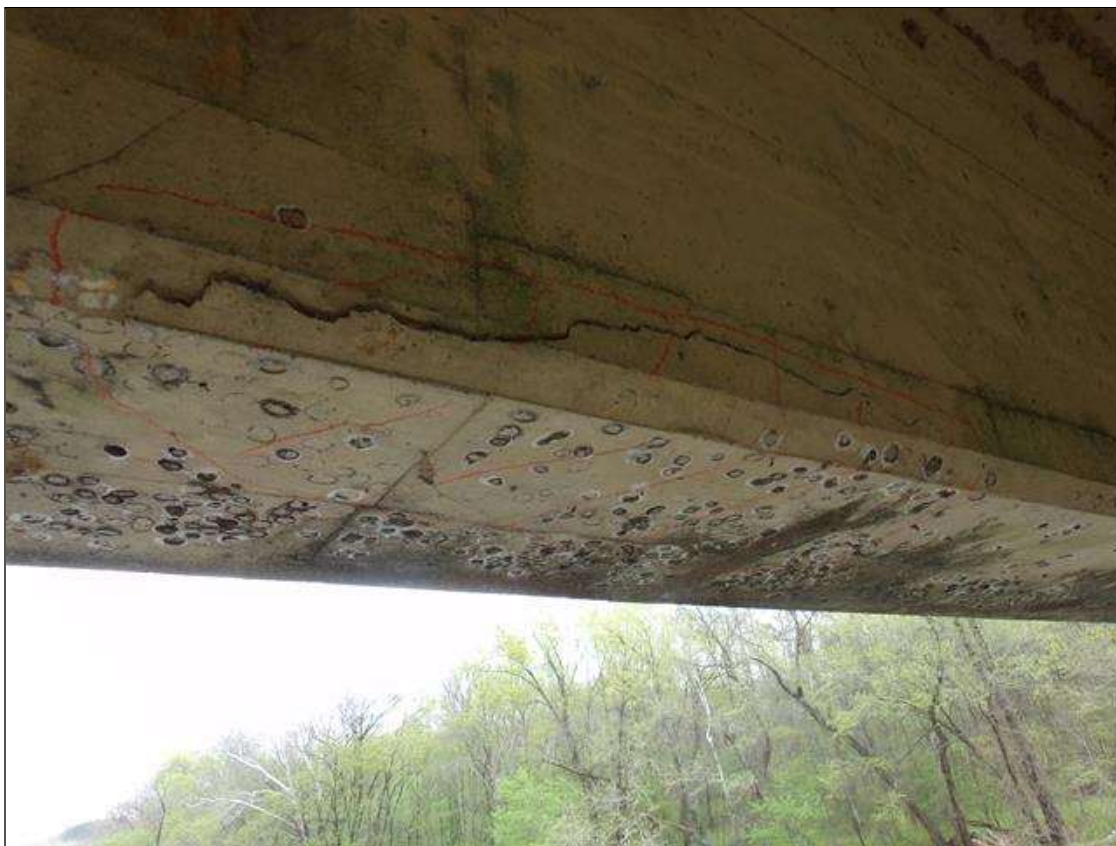
Span 8 Beam 5: Delamination 2' long x 10" wide on bottom of beam x 4" high on west face 10' from pier 7
