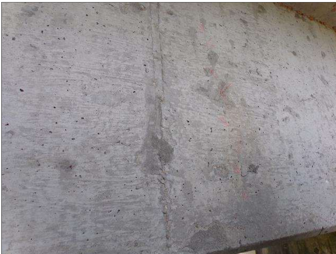
Span 8 Beam 1: Full height vertical hairline to 1/32" crack on west face of beam at mid span.
