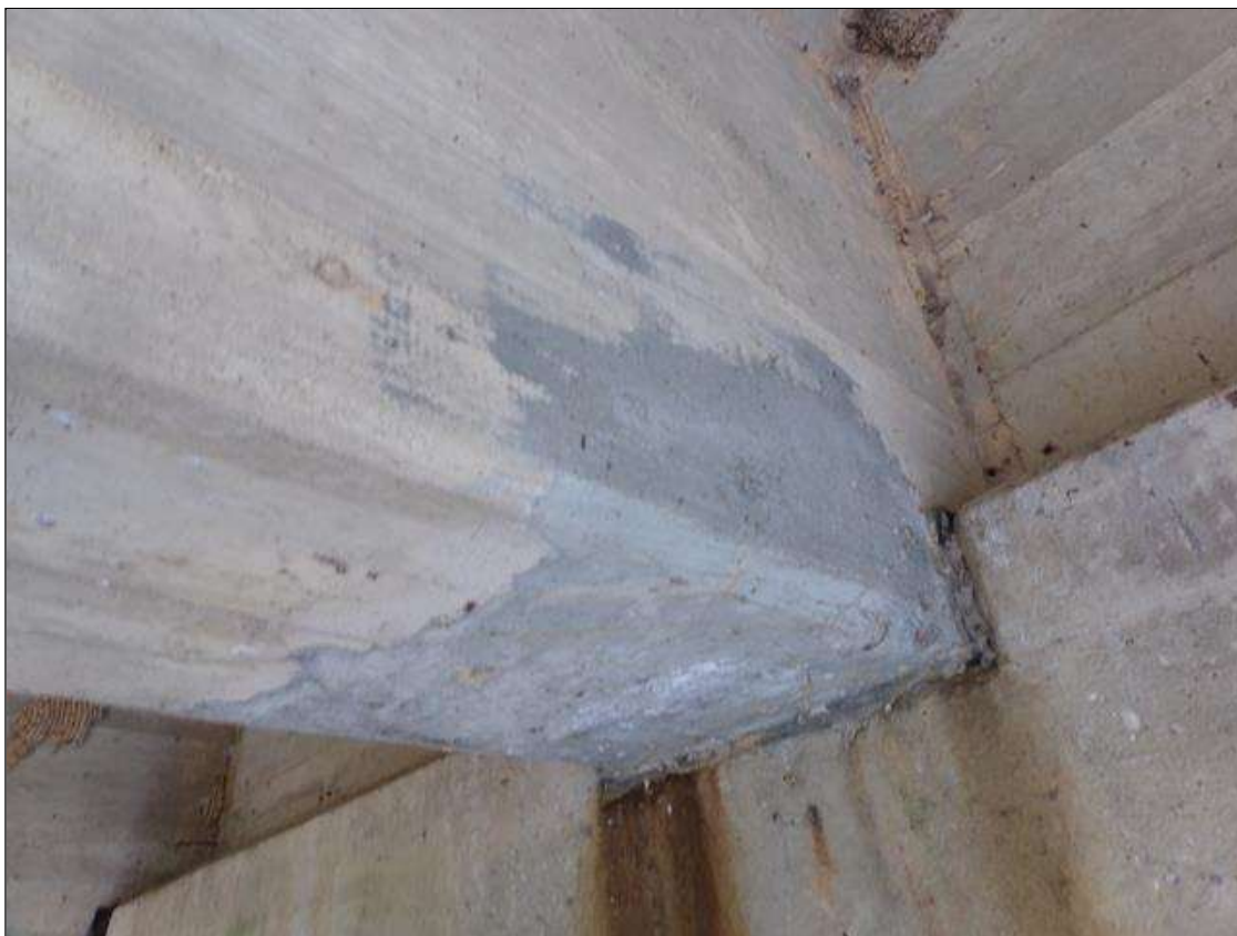
Span 7 Beam 4: Sound patched area 18" long x 1' high on east and west faces of beam at pier 7.
