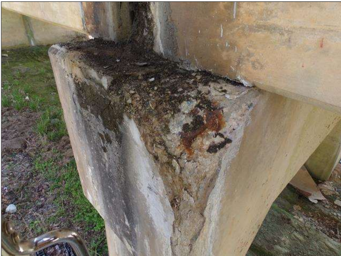
Bent 1 Cap 1: East end is spalled full height on northeast corner 4" wide x 1/4" deep with top corner spalled 16" wide x 12" wide x 2" deep and bottom corner spalled 8" wide x 8" high x 2" deep.
