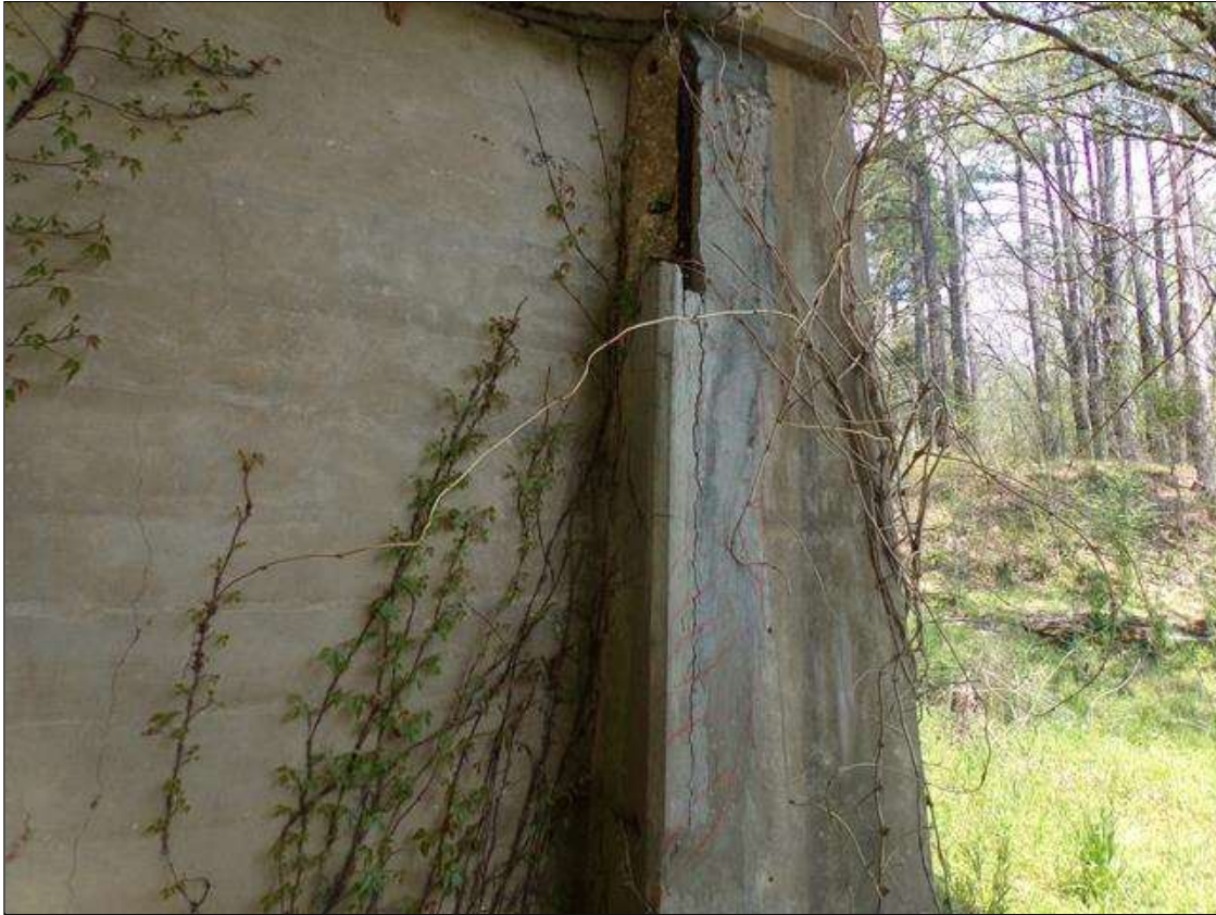
Bent 9 Pile 3: 8' high x up to 1' wide on south face x up to 10" wide on west face delaminated area with spall 3' high x 1' wide x 3" deep with exposed rebar with no measurable section loss starting at bottom of cap.
