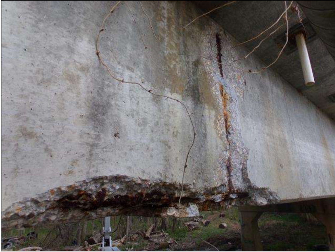
Span 2 Beam 1: Full height spall up to 2' wide x 2" deep with exposed rebar with section loss that extends down to bottom corner spall that is 5' long x up to 1' wide by up to 3" deep with exposed rebar with section loss on west face of beam 3' from pier 2.
