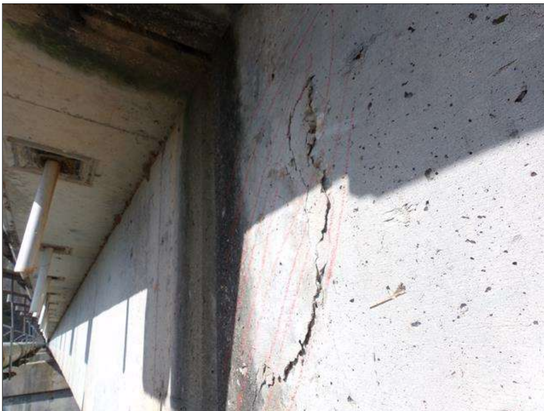
Span 4 Beam 1: Area of delamination 18" wide x 32" high on west face of beam over pier 4
