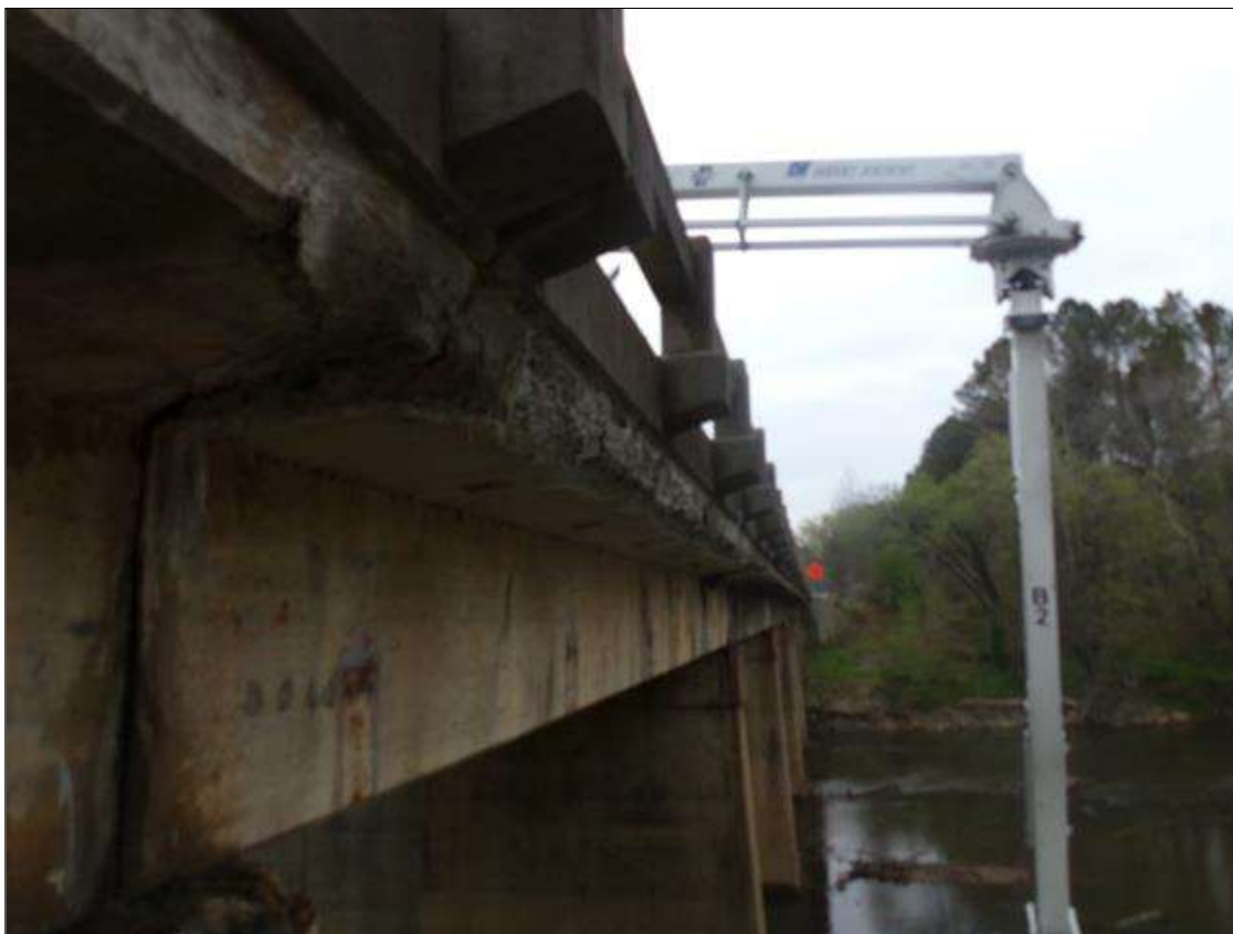
Span 5 Deck: Patched area 1' high x full length of east overhang that is distressed with efflorescence/stalactites/staining and cracking throughout
