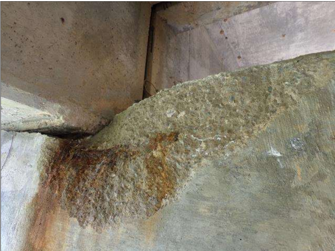
Bent 1 Cap 1: 2' long x 1' wide x 4" deep spall with exposed rebar with no measurable section loss on south face of cap under bay 1.
