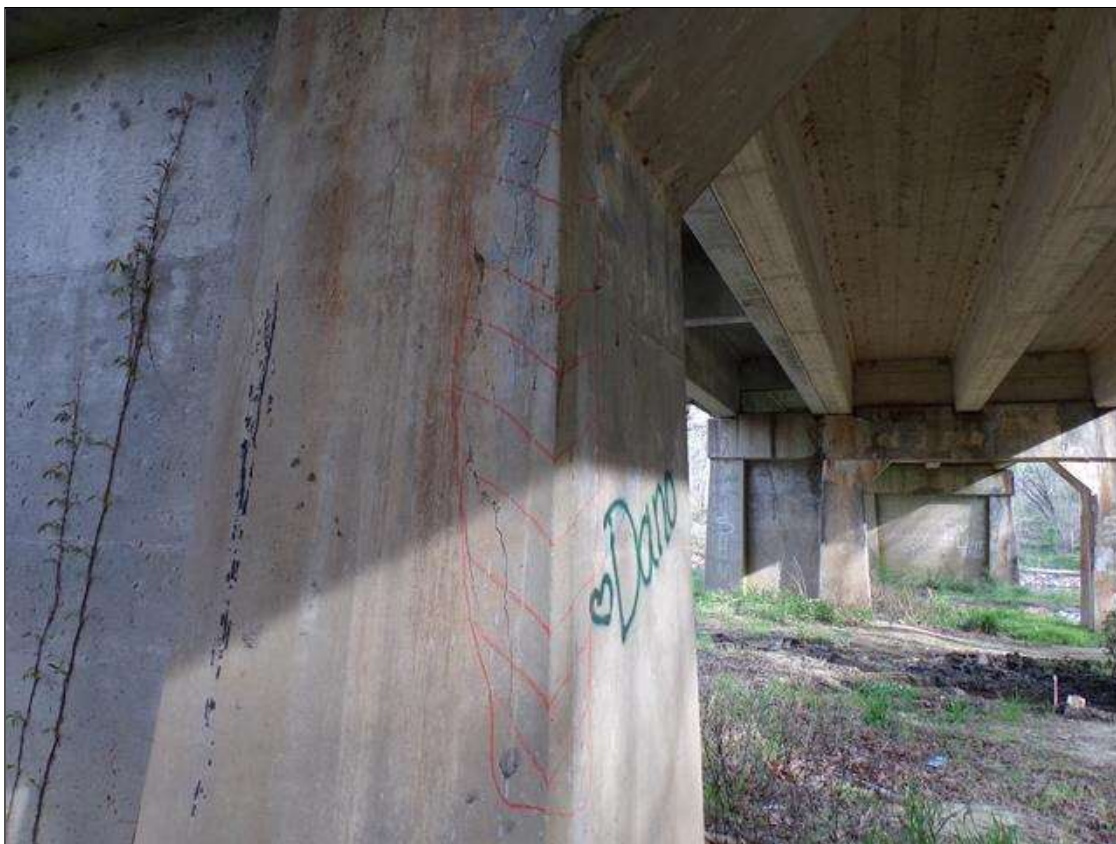
Bent 2 Pile 2: 4.5' high x 16" wide delaminated area on southeast corner starting 2' from bottom of cap.
