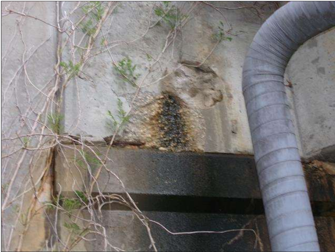
End Bent 2 Abutment/Backwall : 1.5' square area of delamination with a 1.5' square spall x up to 2" deep to the right of delamination with exposed rebar with no measurable section loss starting 3' west of beam 1.
